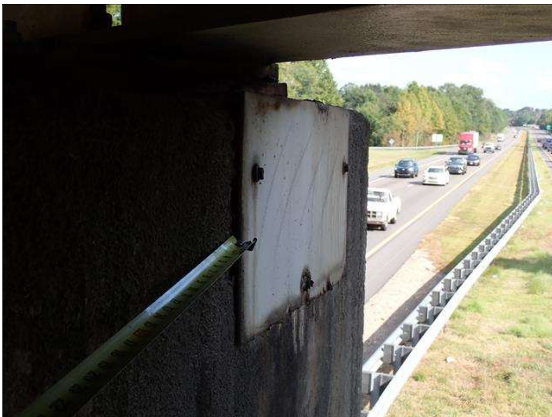
Bent 2 Cap 1: plate repair (25 inch x 11 inch), at south face, under beam 5.
