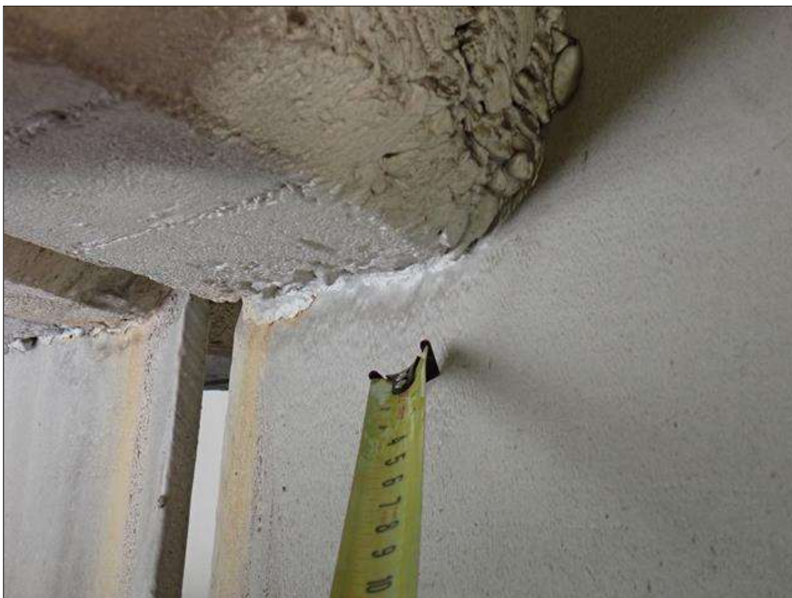
Span 4 Beam 4: (PAR) at bent 3, web adjacent to diaphragm, painted over section loss (5/16 inch average remaining x 10 inch x 1.5 inch)
