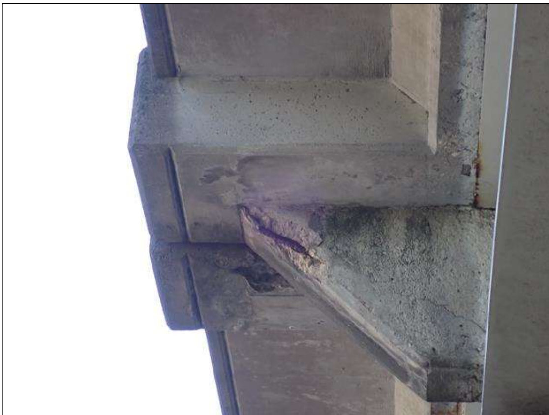
Span 1 Beam 1: 15 inch x 6 inch x 2 inch deep spall with exposed reinforcing in end diaphragm overhang, west side, at bent 1.
