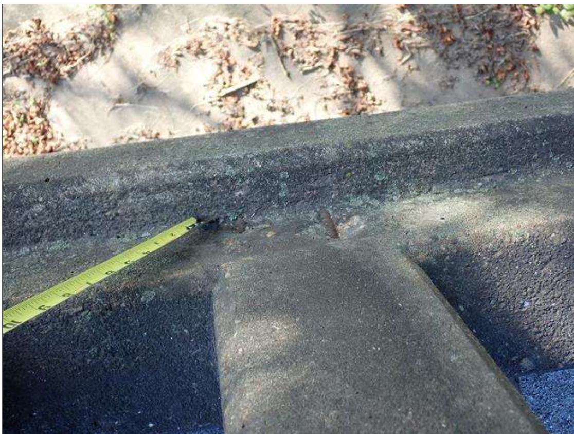
Span 1 Right Bridge Rail: 16 - spalls with exposed reinforcing up to 2 inch x 1 inch x 1/2 inch deep, in outside face, at random.
