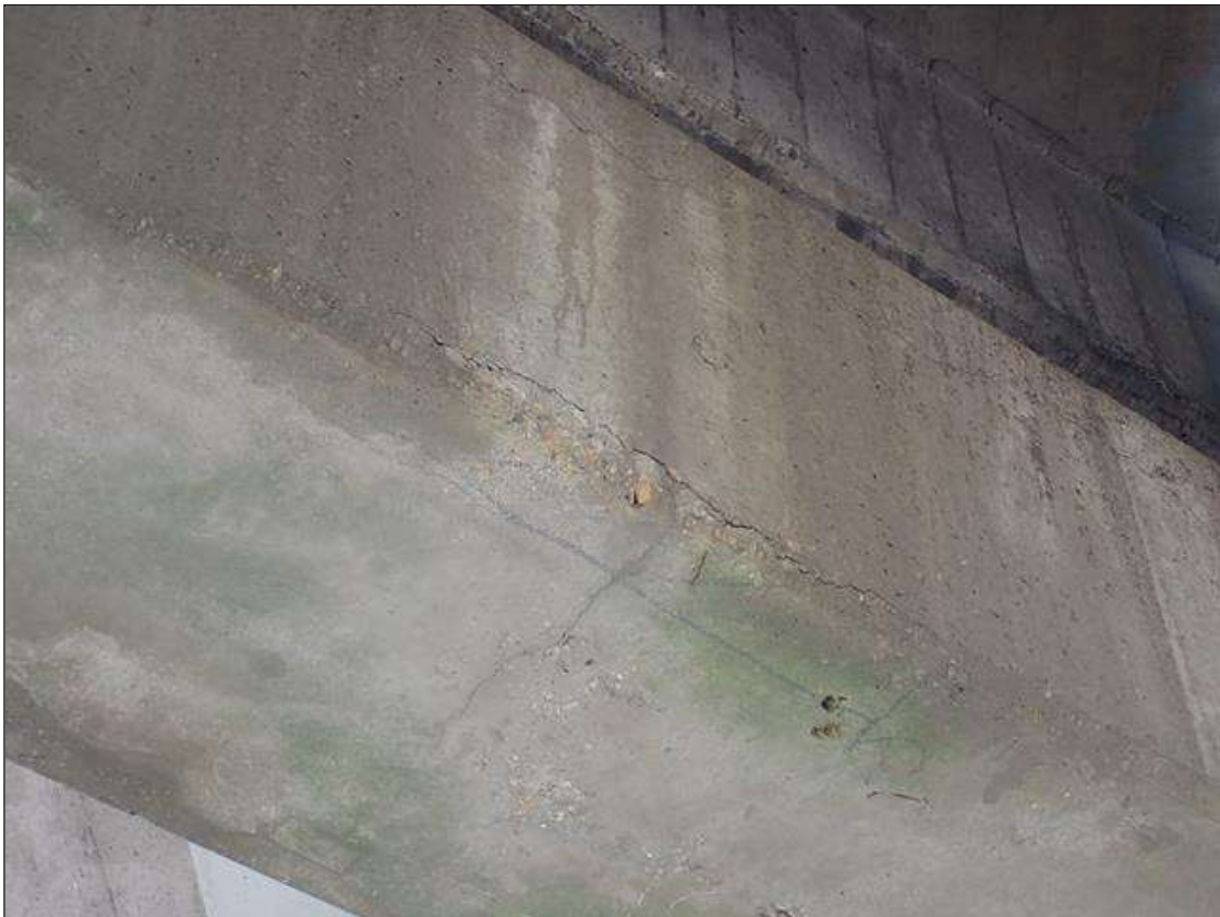
Bent 2 Cap 1: under bay 3 at North face extending to underside, delamination [31 inch x 6 inch] with associated cracks [up to 1/32 inch]
