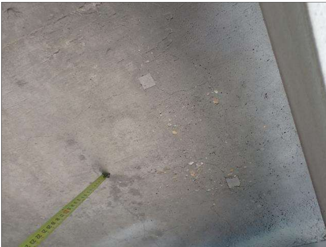
Span 4 Deck: throughout underside of deck, map cracks (hairline) at random
