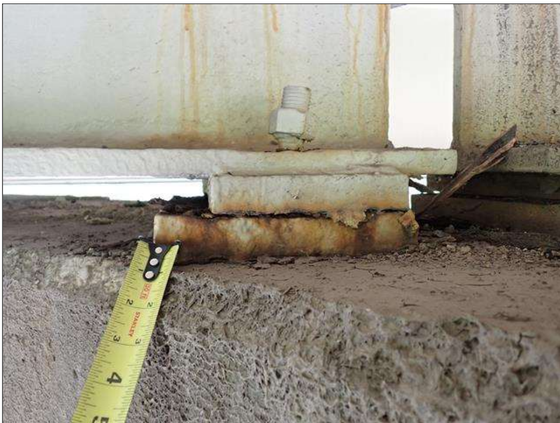
Span 2 Beam 4 - Far Bearing 4: surface rust/pack rust.
