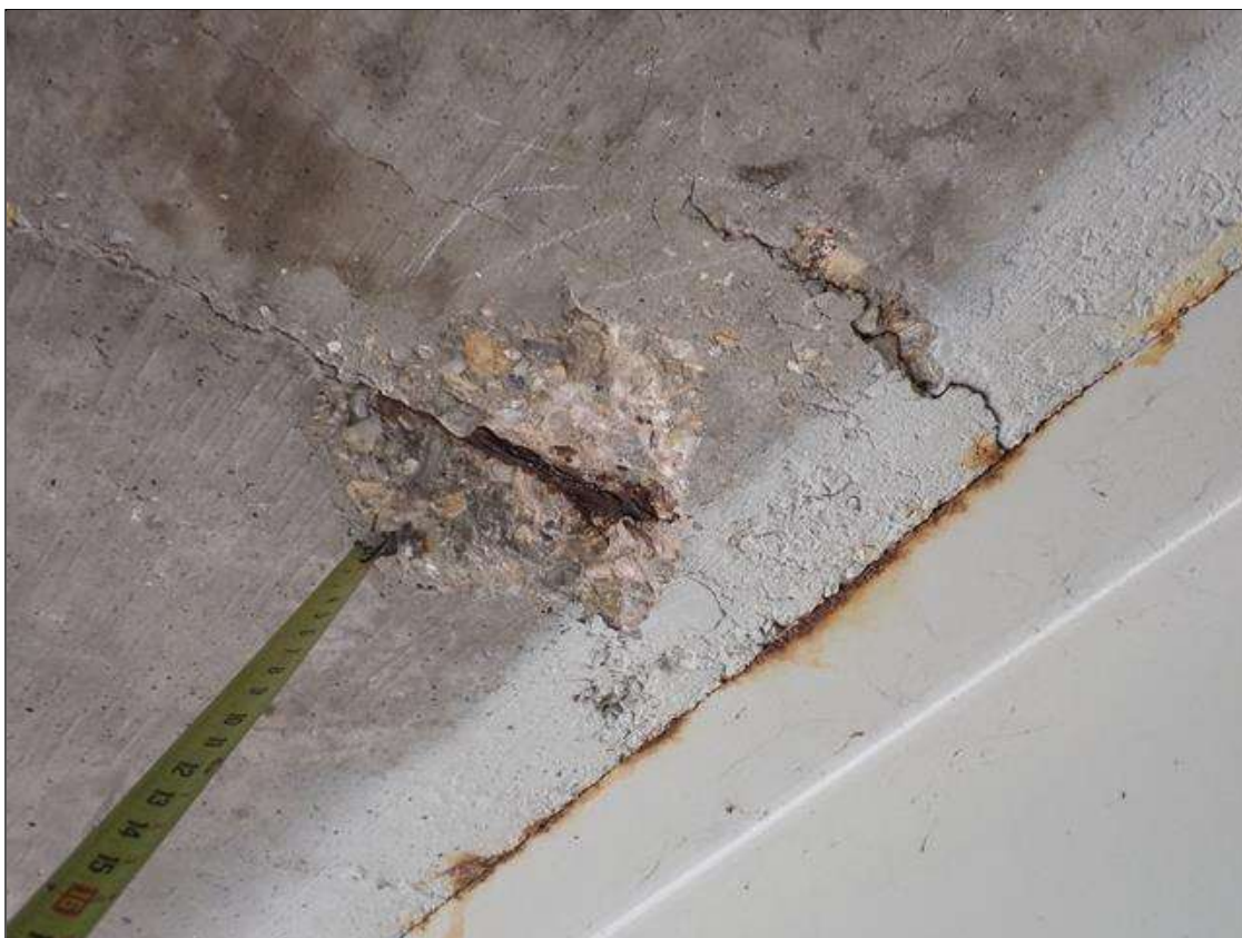
Span 4 Deck: (PAR) bay 1, near end bent 1, spall/delamination (15 inch diameter x 1.5 inch deep) with exposed rusted rebar
