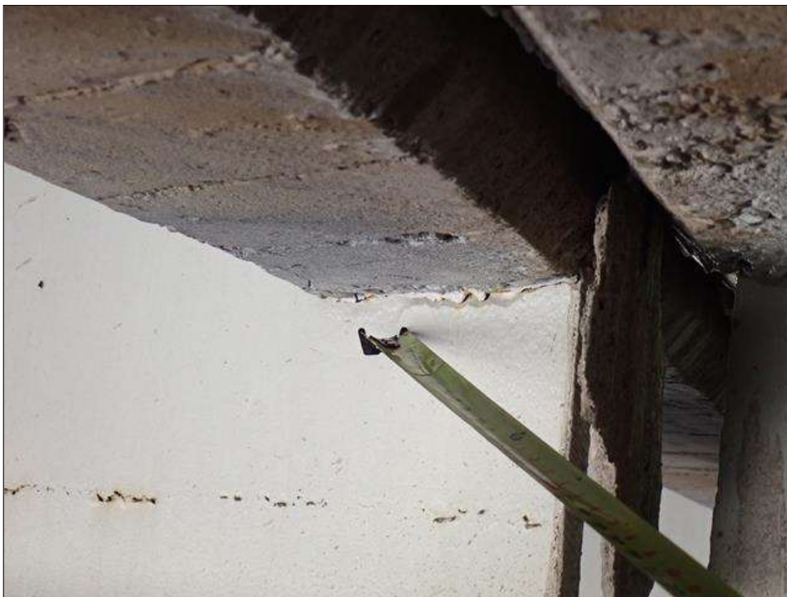
Span 2 Beam 2: at bent 1, web adjacent to diaphragm, painted over section loss (7/16 inch average remaining x 9 inch x 1 inch)
