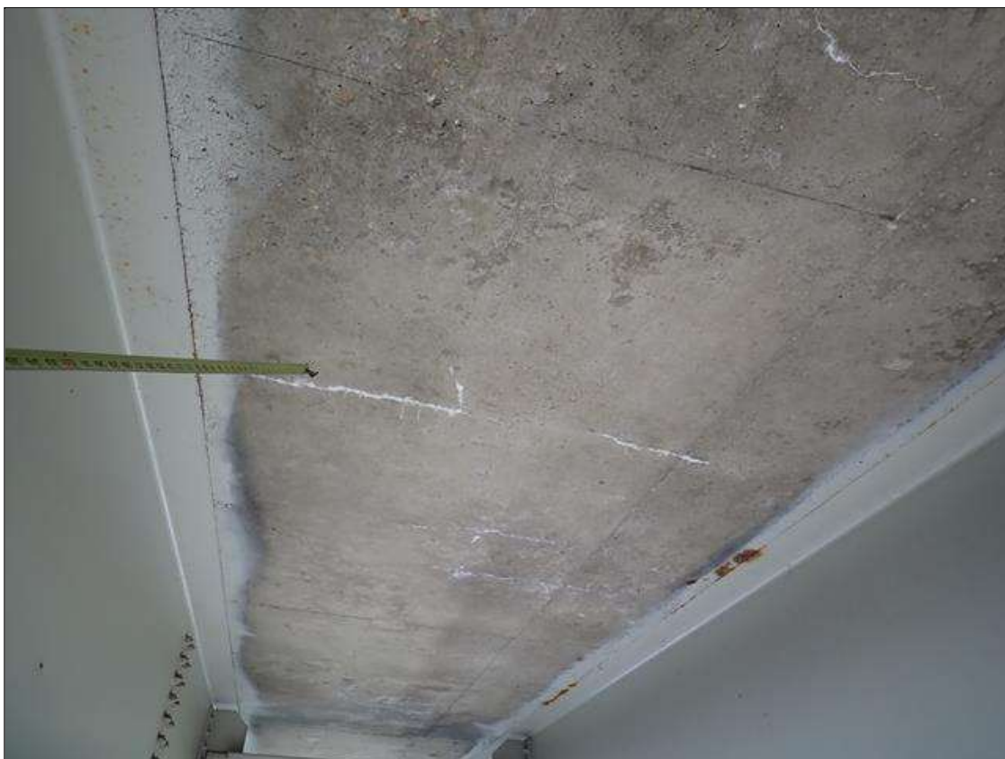
Span 1 Deck: (PAR) underside of all bays, transverse and map cracks (up to 1/32 inch) with efflorescence buildup and some rust stains at random
