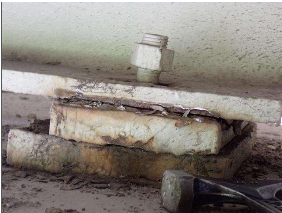
Span 2 Beam 2 - Far Bearing 2: (PAR) along east face, between sole plate and bottom flange, broken weld; right anchor bolt nut backed off
