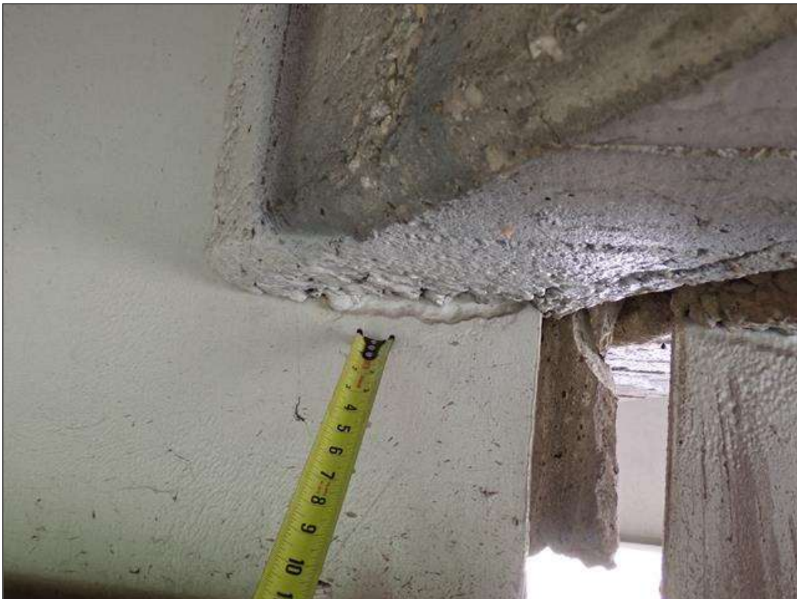
Span 1 Beam 2: (PAR) at bent 1, web adjacent to diaphragm, painted over section loss (1/4 inch average remaining x 10 inch x 2 inch)
