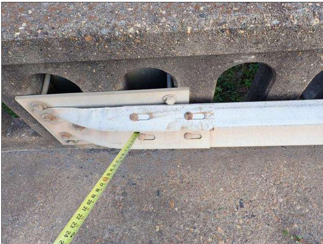
(PAR) northwest guardrail attachment, improper lap
