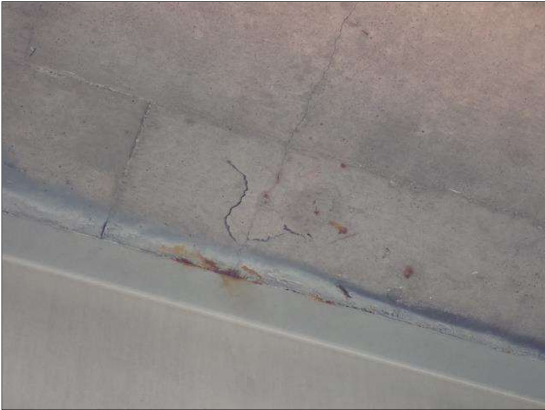
Span 3 Deck: [PAR] 19 inch x 16 inch area of delamination on underside of deck in bay 1, over left shoulder
