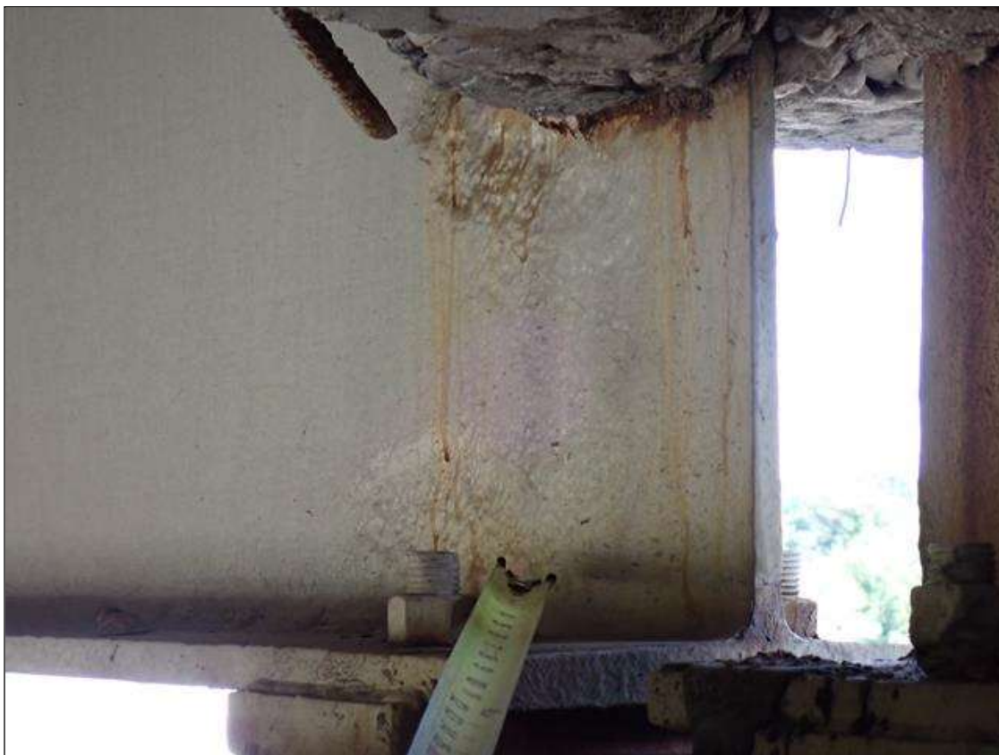
Span 3 Beam 5: (PAR) at bent 2, painted over section loss: web adjacent to diaphragm (3/8 inch average remaining x 8 inch x 4 inch); lower web (3/8 inch average remaining x 10 inch x 5 inch) with corrosion reinitiated
