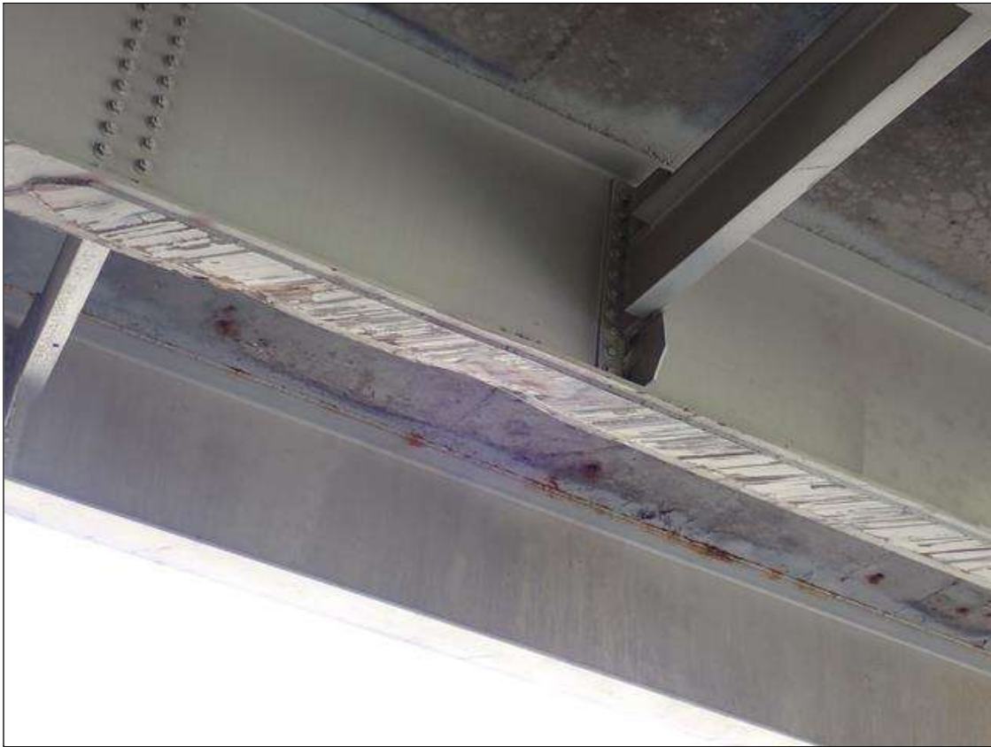
Span 2 Beam 2: (PAR) over both travel lanes, underside of bottom flange and cover plate, impact scrapes with gouges (up to 1/2 inch deep); over right travel lane, bottom flange and cover plate, distorted (up to 1 inch upwards x approximately 1.5 feet); no apparent distress to cover plate welds
