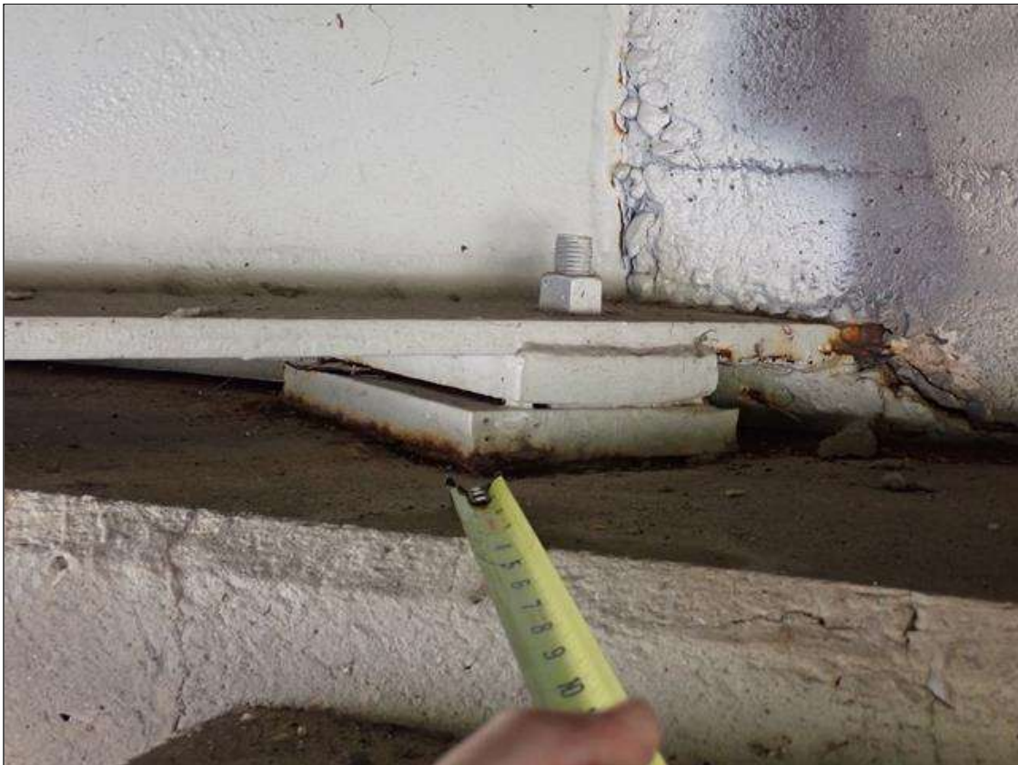
Span 1 Beam 3 - Near Bearing 3: surface rust
