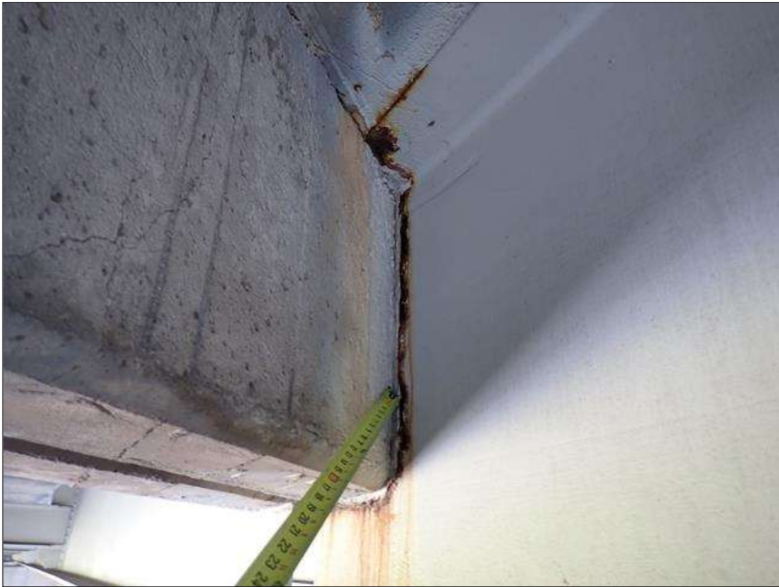
Span 2 Beam 3: at bent 2, corrosion with section loss: web adjacent to diaphragm (7/16 inch x 10 inch x up to 2 feet); top flange (3/4 inch average remaining x 3 inches)
