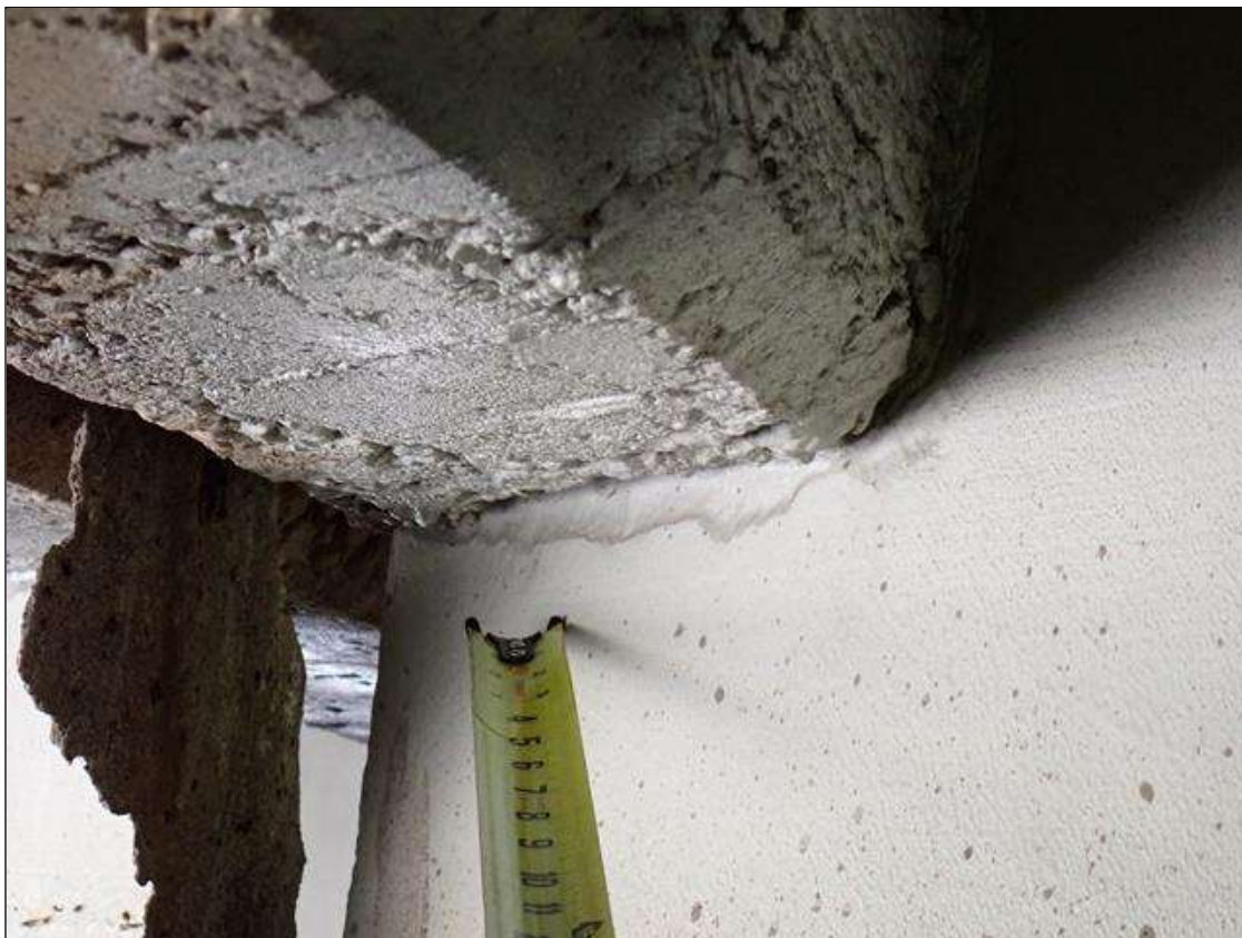
Span 1 Beam 2: (PAR) at bent 1, web adjacent to diaphragm, painted over section loss (1/4 inch average remaining x 10 inch x 2 inch)
