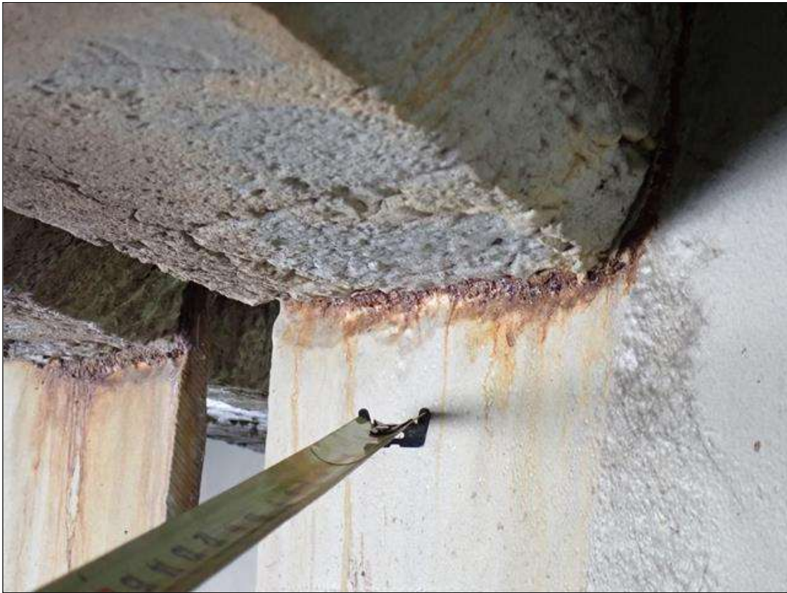
Span 1 Beam 3: (PAR) at bent 1, web adjacent to diaphragm, painted over section loss (5/16 inch average remaining x 10 inch x 1 inch) with adjacent painted over pitting (up to 1/8 inch deep x 2 inch x 3 inch) with corrosion reinitiated
