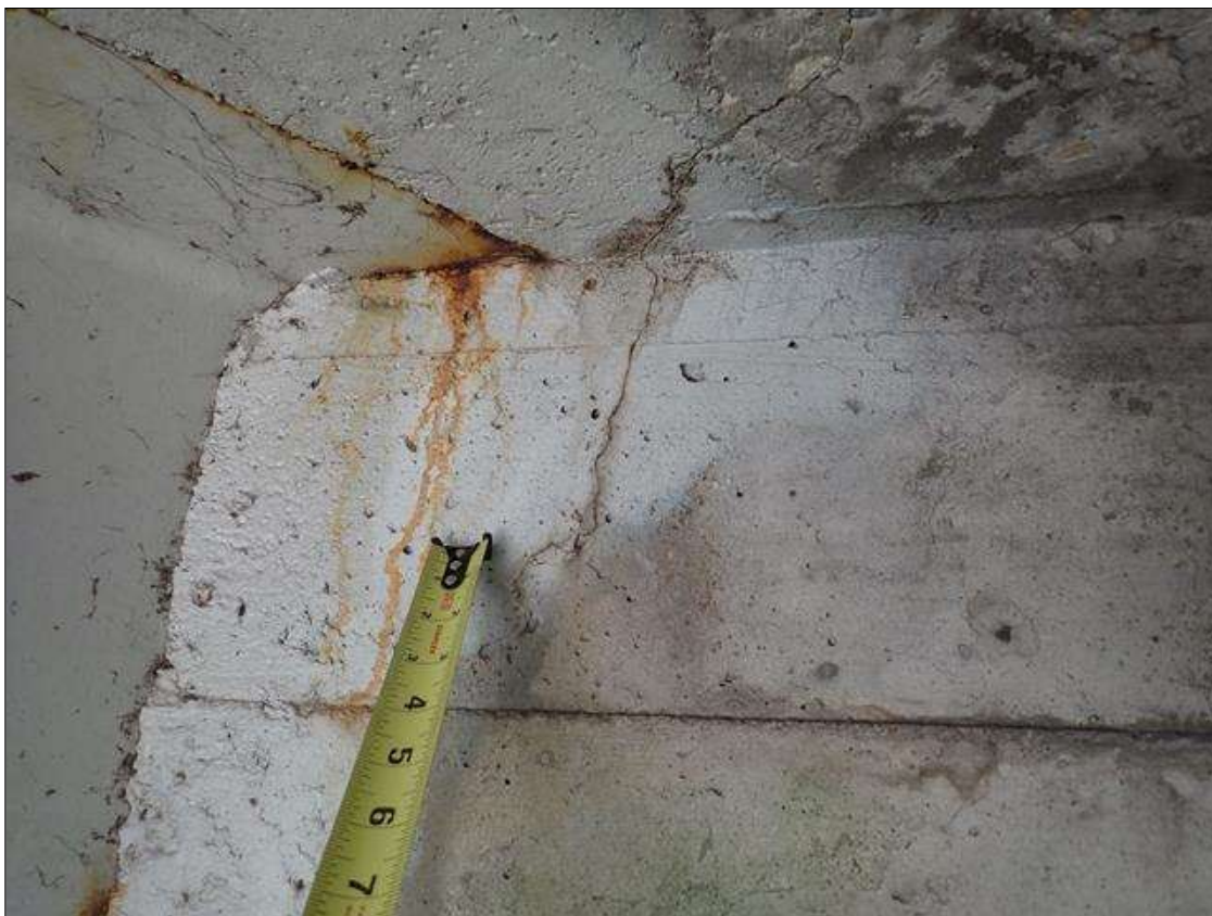
End Bent 2 Abutment: along the length of the abutment, vertical cracks (up to 1/32 inch x 1 foot) and areas of map cracks (hairline) at random
