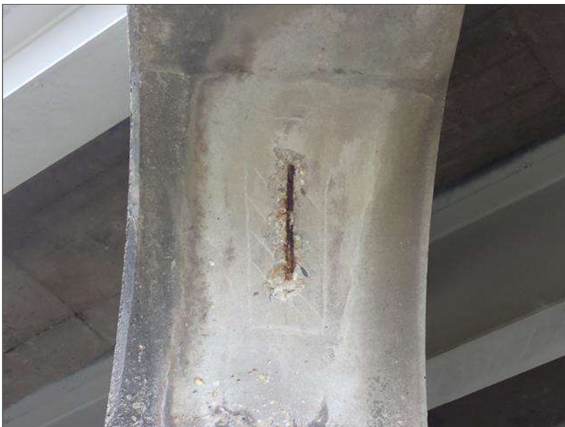
Bent 2 Cap 1: 1 foot x 3 inch x 1/2 inch deep spall with exposed reinforcing [no measurable section loss], underside of east end of overhang.
