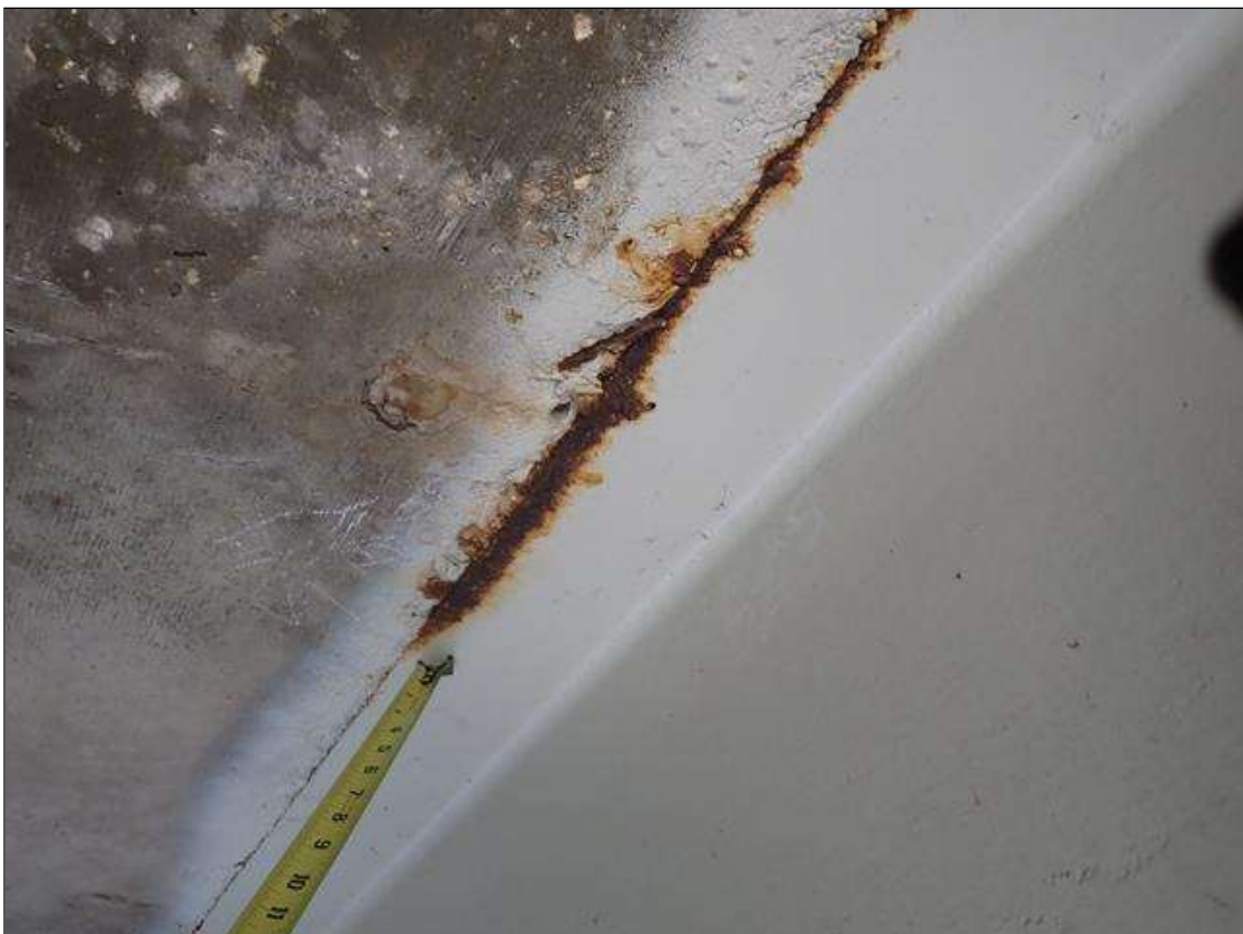
Span 4 Beam 5: surface rust along edge of top flange, on west side, and along east face of web, at random.
