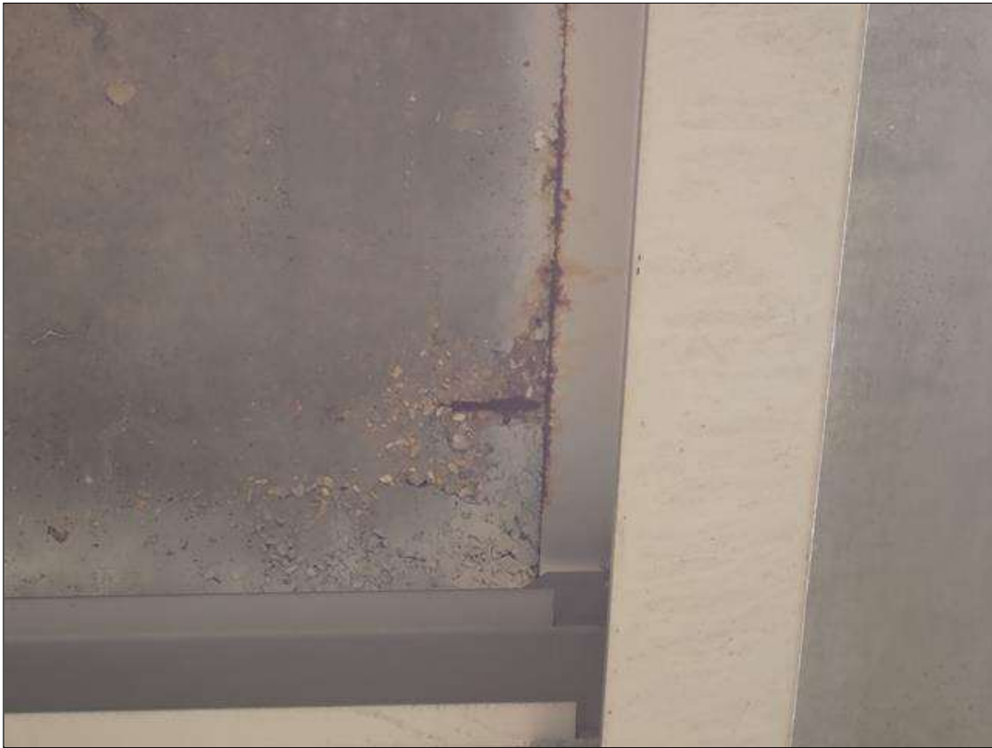
Span 4 Deck: (PAR) bay 4, near midspan, spall (10 inch diameter x 1.5 inch deep) with exposed rusted rebar
