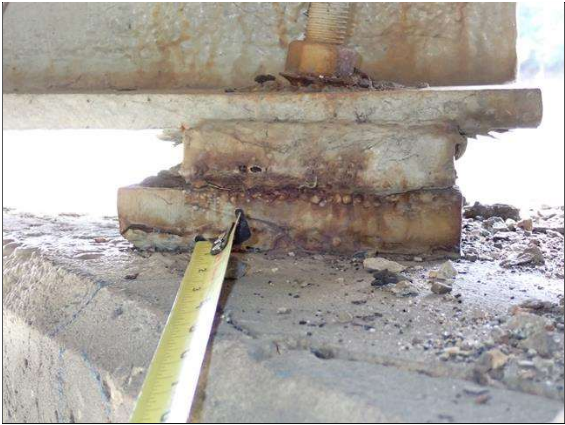
Span 4 Beam 5 - Near Bearing 5: surface rust/pack rust.
