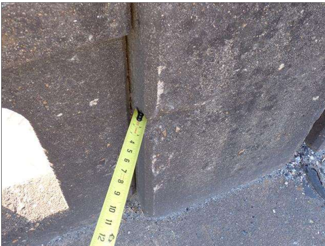
Span 4 Right Bridge Rail: 4 inch x 4 inch x 1.5 inch deep spall, in traffic face, at bent 3.
