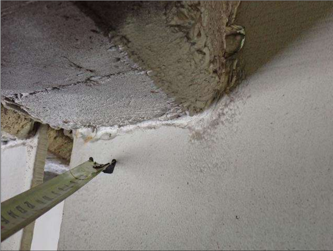
Span 4 Beam 2: (PAR) at bent 3, web adjacent to diaphragm, painted over section loss (3/8 inch average remaining x 10 inch x 1 inch)
