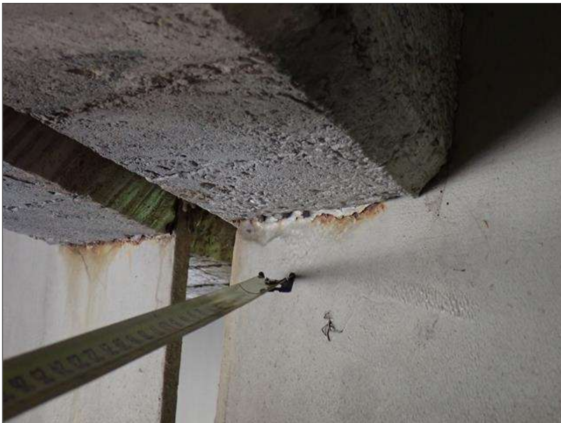
Span 1 Beam 4: (PAR) at bent 1, web adjacent to diaphragm, painted over section loss (3/8 inch average remaining x 7 inch x 1 inch) with corrosion reinitiated
