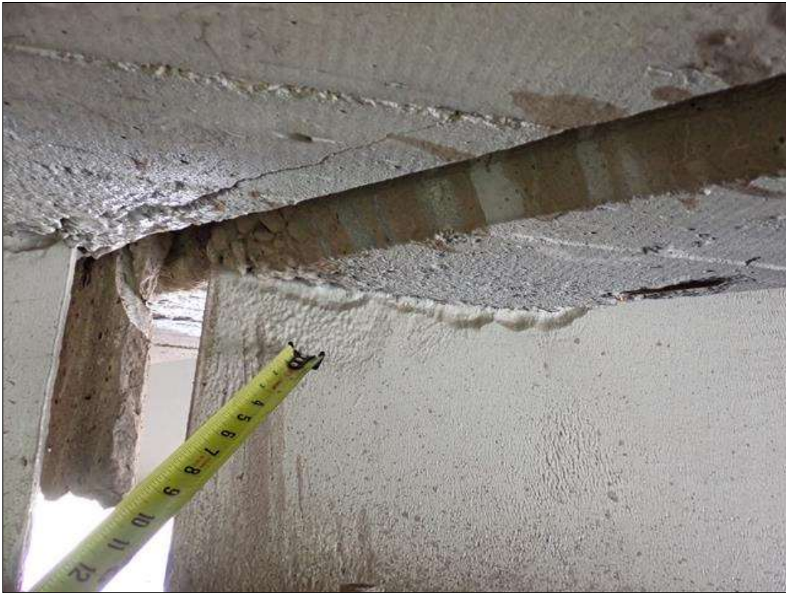
Span 2 Beam 2: (PAR) at bent 1, web adjacent to diaphragm, painted over section loss (5/16 inch average remaining x 9 inch x 1 inch)
