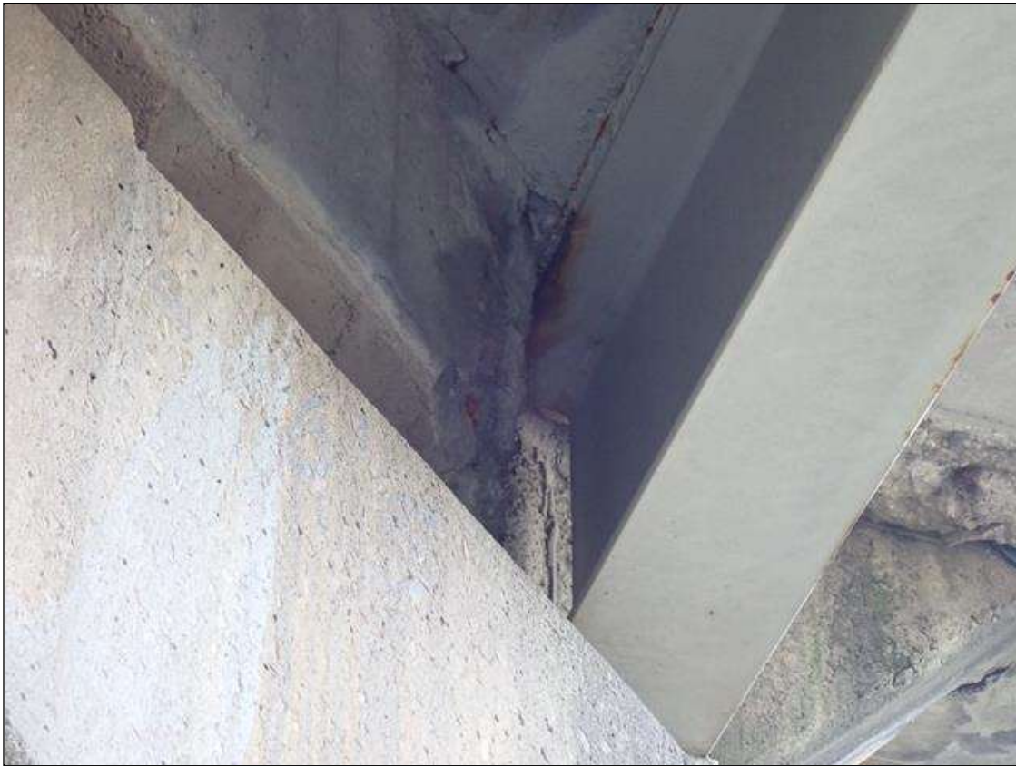
Span 2 Beam 1: end diaphragm on both sides has been removed with exposed rusted rebar, at both ends, when beam was replaced.
