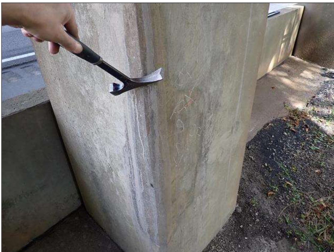
Bent 1 Pile 2: 6 foot x 18 inch sound patch at southwest corner, near base of column.
