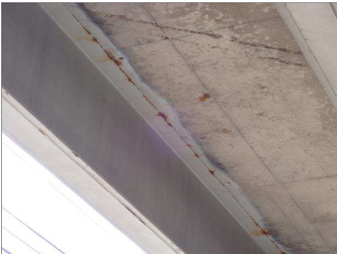
Span 3 Beam 5: along the length of the beam, along edges of top flange, at random
