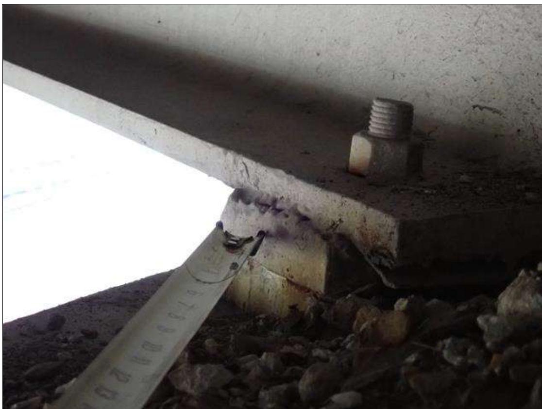
Span 3 Beam 3 - Near Bearing 3: (PAR) west face, between sole plate and bottom flange, poor quality weld with voids
