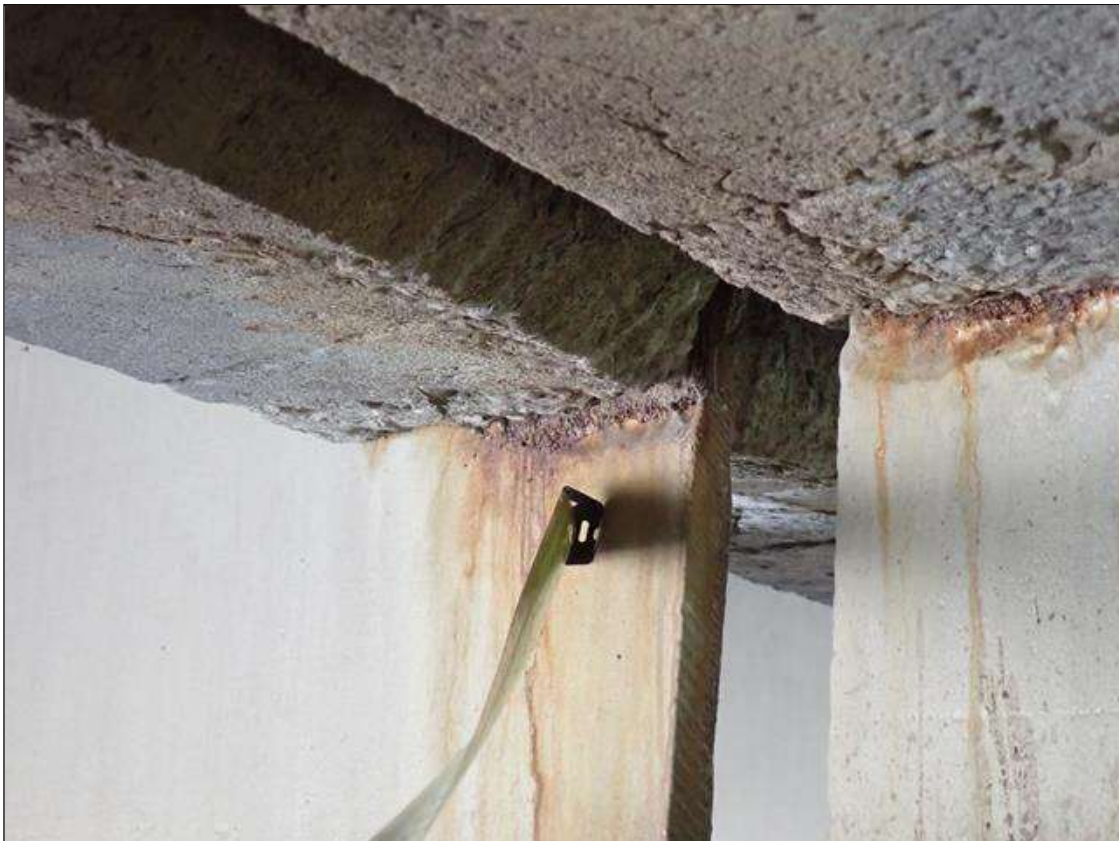
Span 2 Beam 3: (PAR) at bent 1, web adjacent to diaphragm, painted over section loss (5/16 inch average remaining x 6 inch x 1 inch); lower web, painted over pitting (up to 1/8 inch deep x 14 inch x 3 inch) with corrosion reinitiated
