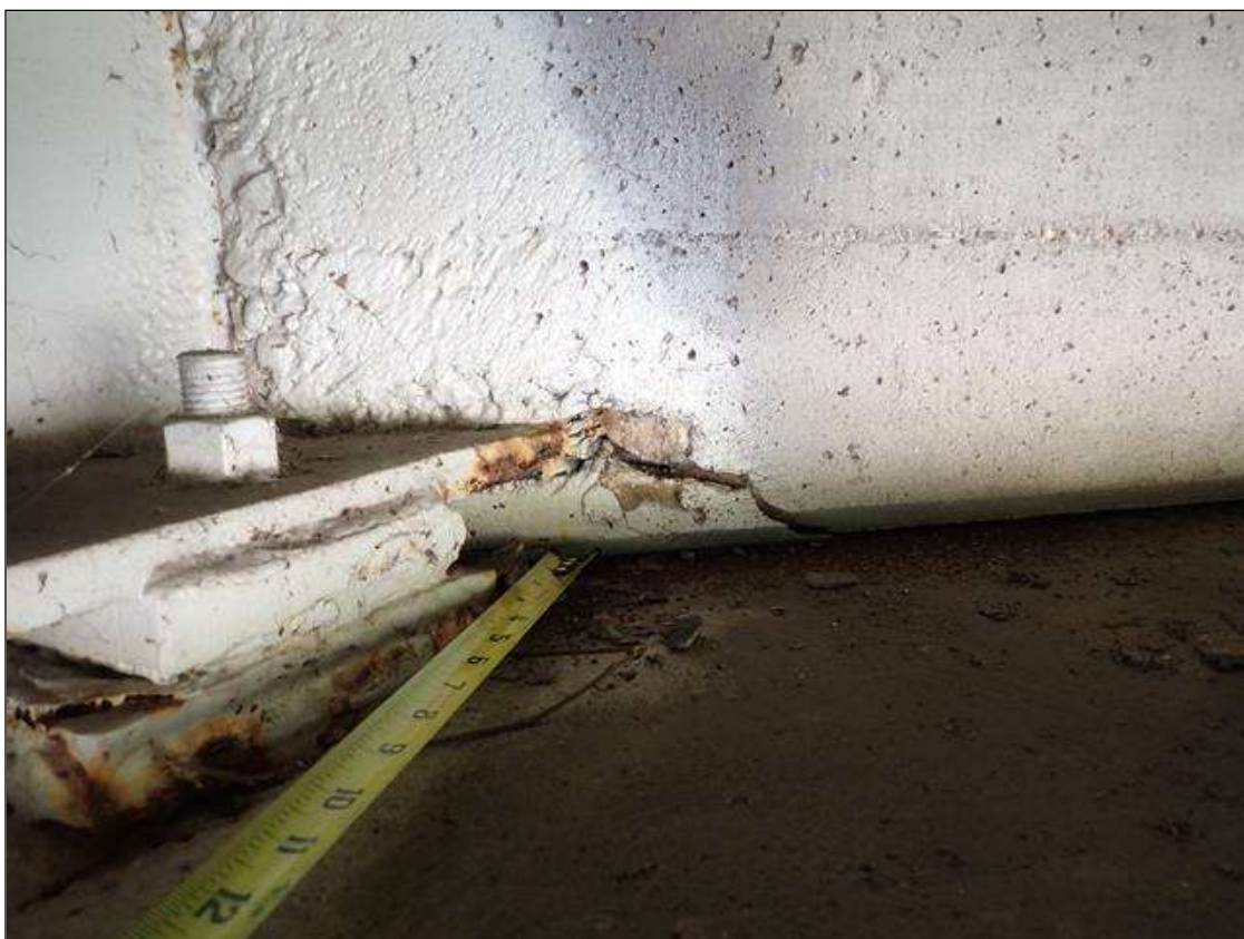
End Bent 1 Abutment: 6 inch x 2 inch delamination with crack up to 1/4 inch wide, left side of beam 3 (similar at all beams).
