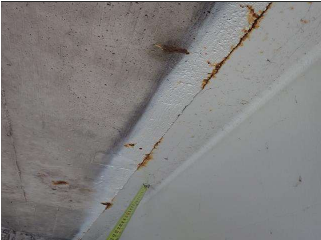
Span 1 Beam 3: near end bent 1 and bent 1, both flanges and web, surface rust at random
