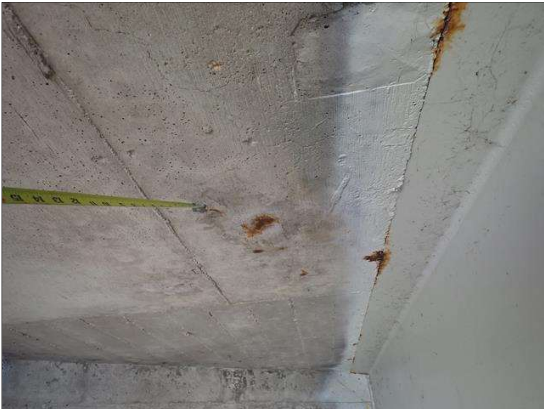
Span 1 Deck: (PAR) underside of all bays, transverse and map cracks (up to 1/32 inch) with efflorescence buildup and some rust stains at random
