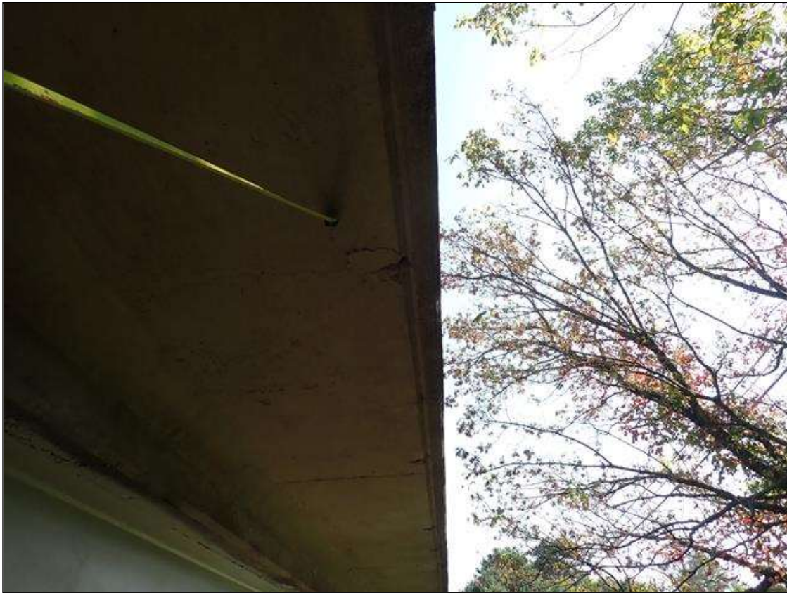
Span 1 Deck: (PAR) both overhangs, delaminations/spalls (up to 4 inch diameter x 1/2 inch deep) with exposed rusted rebar at random
