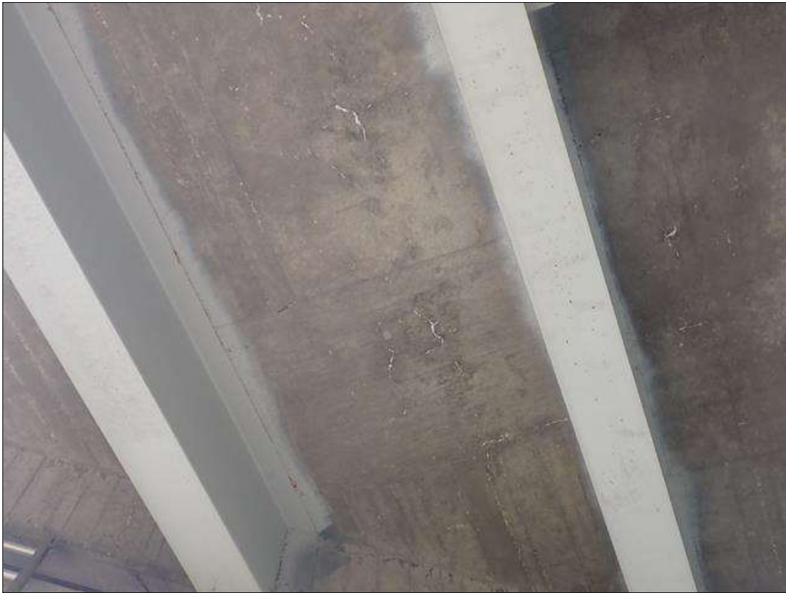
Span 4 Deck: (PAR) underside of all bays, near bent 3 and end bent 2, transverse cracks (up to 1/32 inch x full width) and map cracks (hairline) with efflorescence buildup and some rust stains at random
