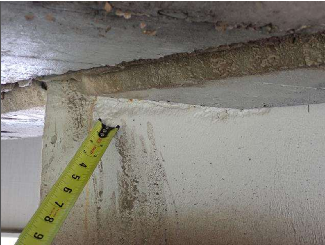
Span 3 Beam 2: (PAR) at bent 3, web adjacent to diaphragm, painted over section loss (7/16 inch average remaining x 4 inch x 1 inch)
