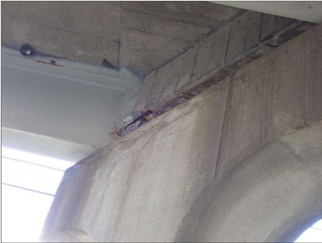
Bent 2 Cap 1: at North face and extending to top face between beam 3 to beam 5, delaminations [up to 6 feet x 1 foot] with associated cracks [up to 1/16 inch]
