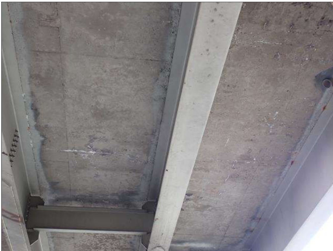
Span 2 Deck: (PAR) throughout underside of deck, in all bays, transverse cracks (up to 1/32 inch x full width) and areas of map cracks (hairline) with efflorescence buildup and some rust stains
