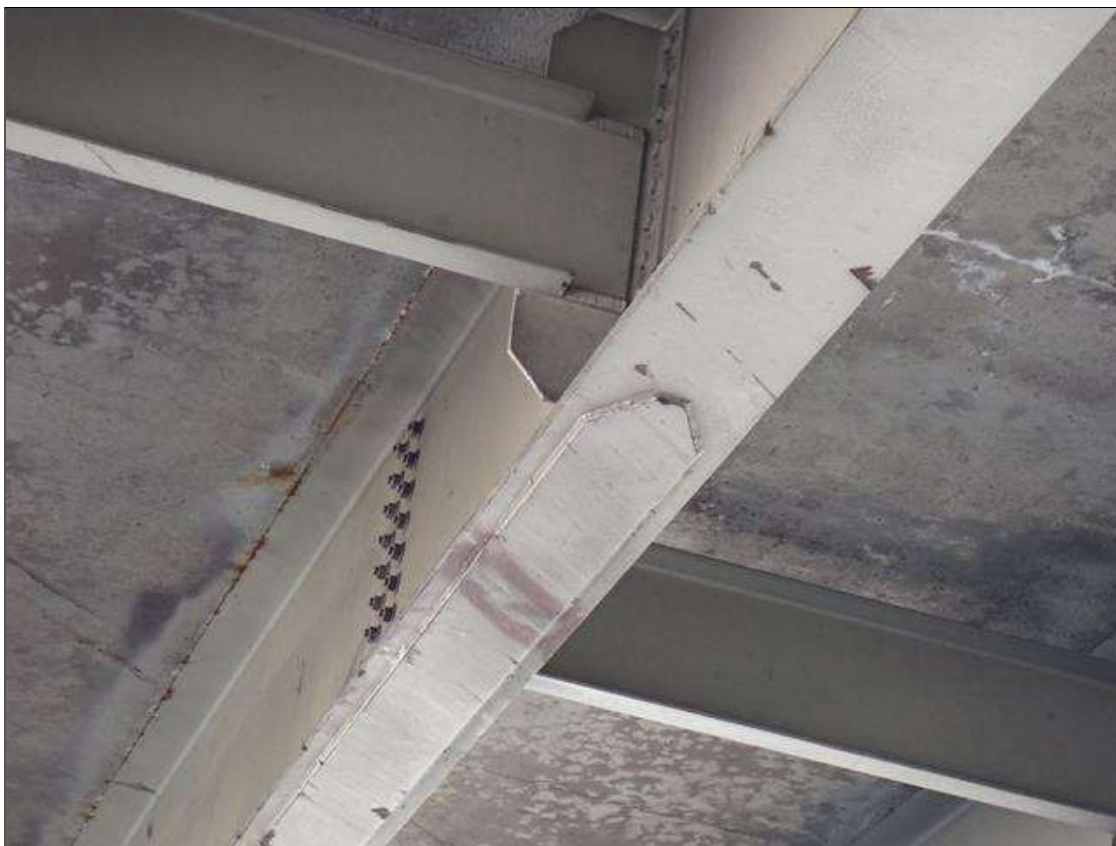
Span 2 Beam 3: over right travel lane, underside of bottom flange and cover plate, impact scrapes with surface gouges; left edge of bottom flange, distorted upwards (approximately 1/4 inch x 8 inches)
