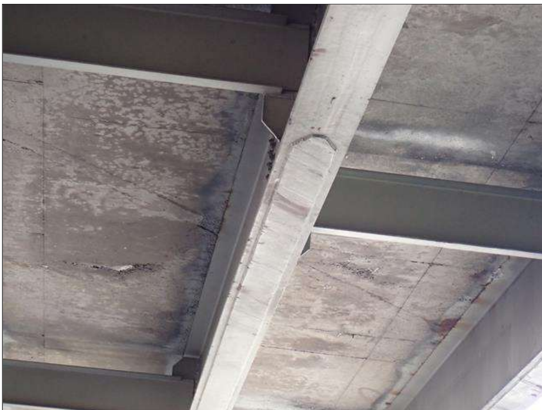
Span 2 Beam 4: over right travel lane, bottom flange and cover plate, impact scrapes with surface gouges
