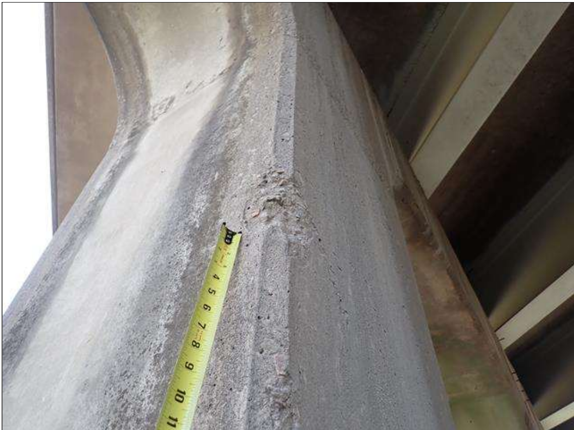
Bent 2 Pile 1: 6 inch x 4 inch x 1 inch deep spall, at southwest corner, 8.5 feet above ground.
