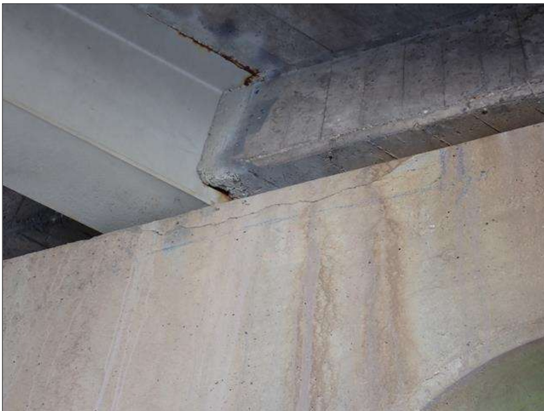
Bent 1 Cap 1: north face, below beam 3, delamination (3 feet x 6 inch) with associated cracks (up to 1/32 inch)
