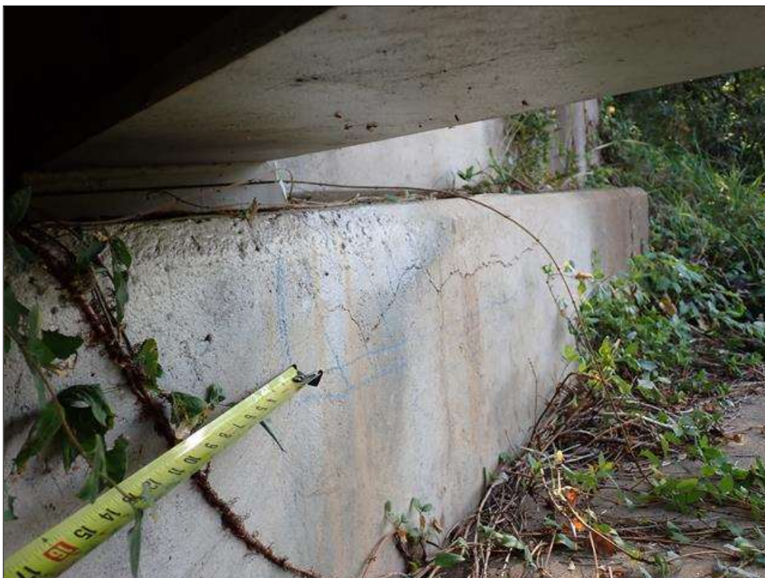
End Bent 2 Cap 1: 4 foot x 8 inch delamination with associated cracks up to 1/16 inch, face of cap, under beam 5.
