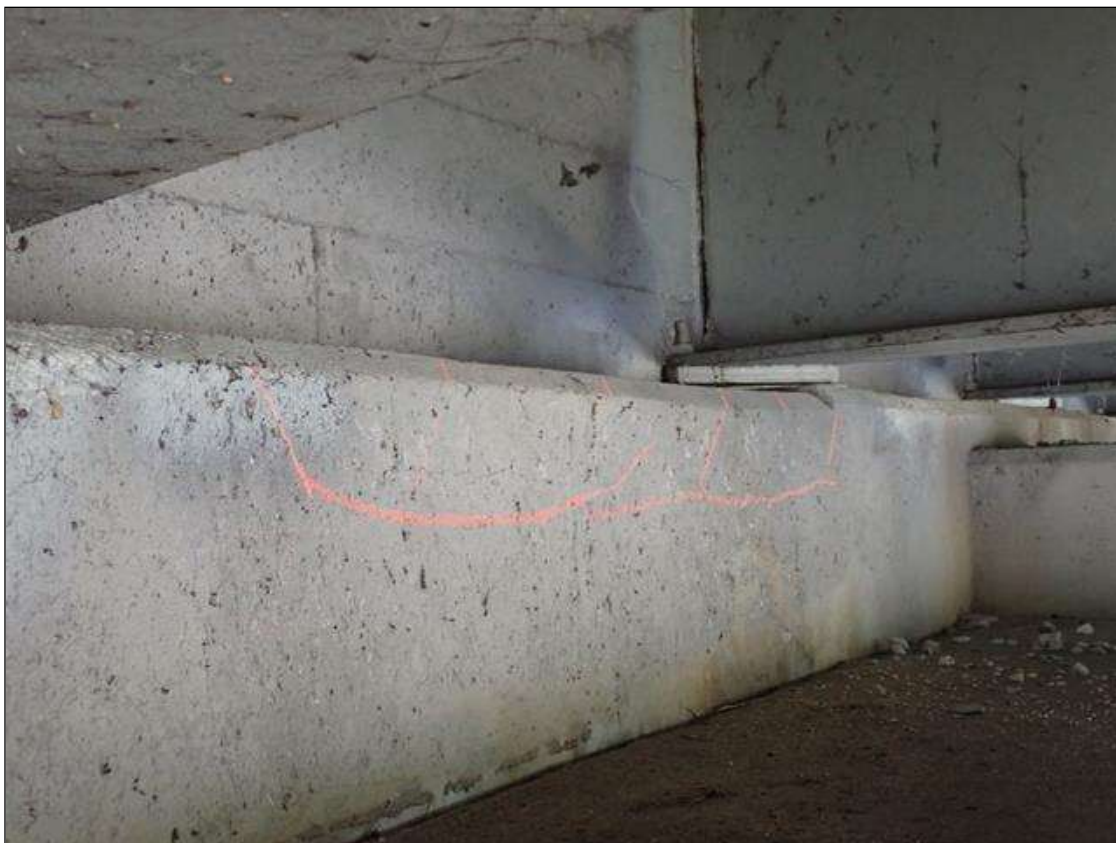
End Bent 1 Cap 1: under bays 3 and 4 on both faces, delaminations [up to 5.5 feet x up to 16 inch] with cracks [up to 1/16 inch]
