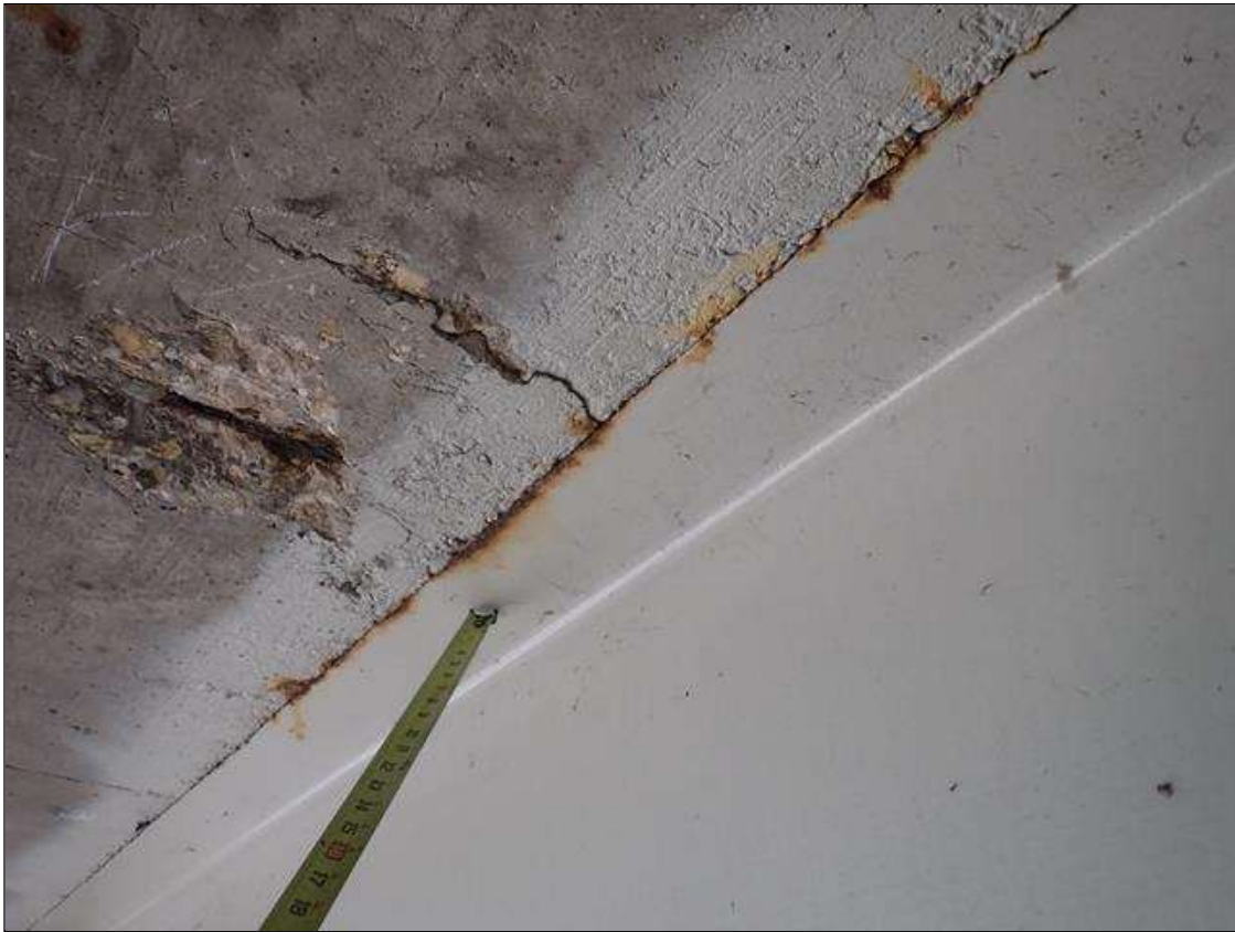
Span 4 Beam 1: near bent 3 and end bent 2, both flanges and web, surface rust at random
