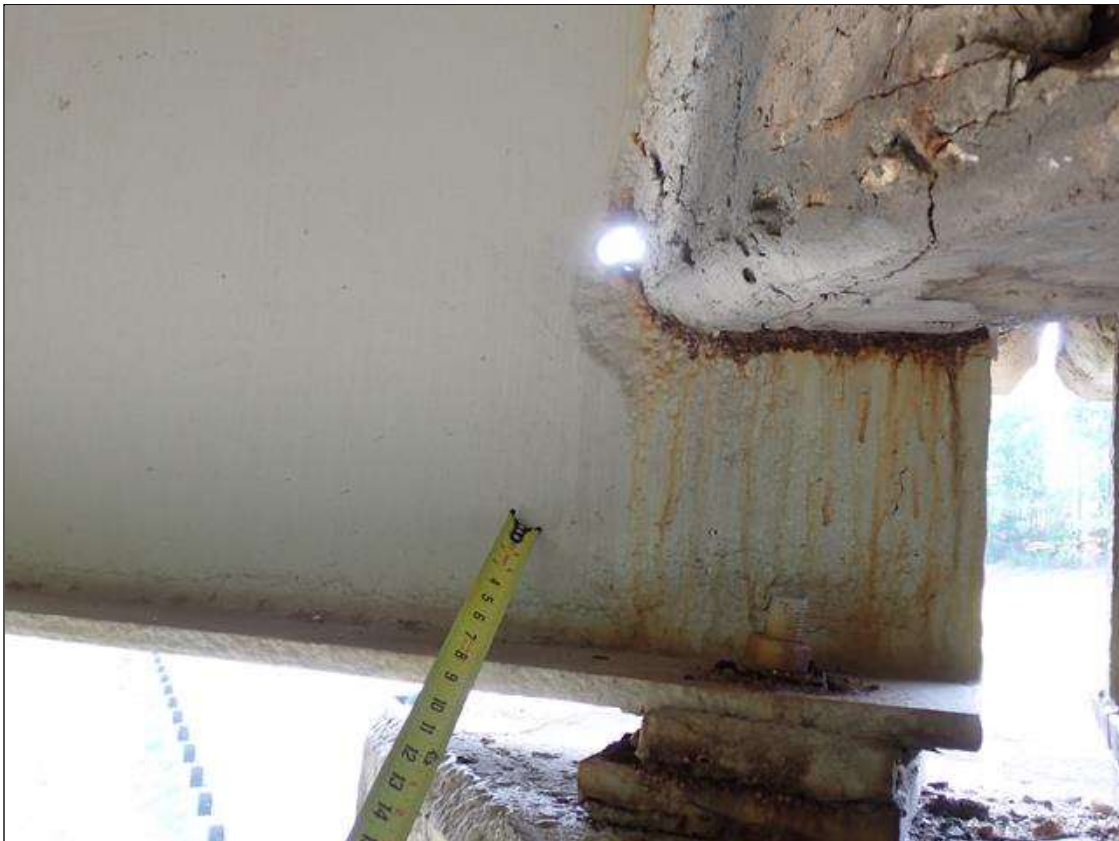
Span 4 Beam 5: (PAR) at bent 3, painted over section loss: web adjacent to diaphragm (1/4 inch average remaining x 10 inch x 4 inch); lower web (3/8 inch average remaining x 2.5 feet x 4 inches with corrosion reinitiated)
