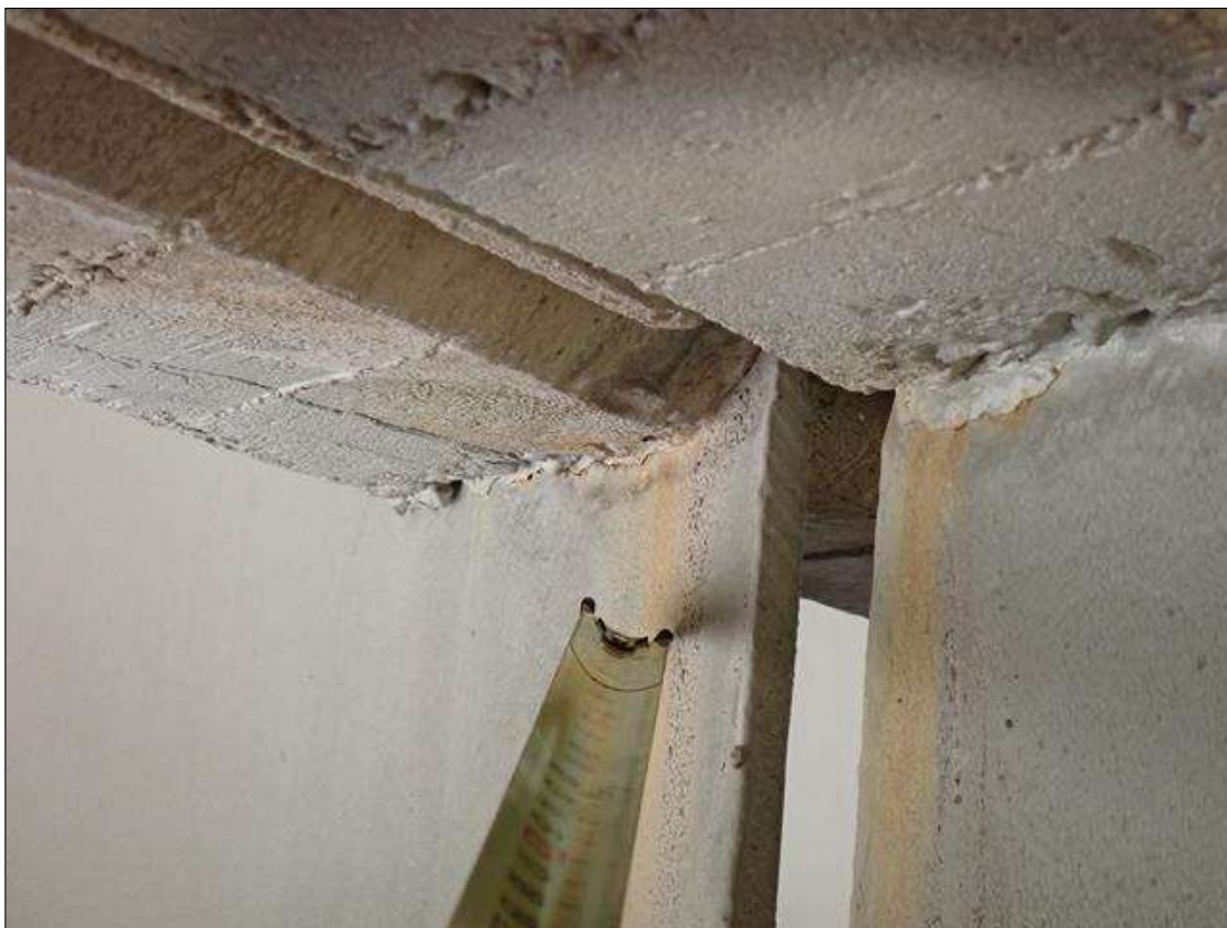
Span 3 Beam 4: (PAR) at bent 3, web adjacent to diaphragm, painted over section loss (5/16 inch average remaining x 5 inch x 1 inch)
