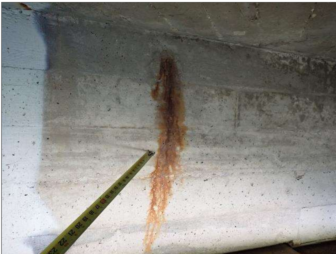
End Bent 1 Abutment: (PAR) area of rust staining in bay 1.
