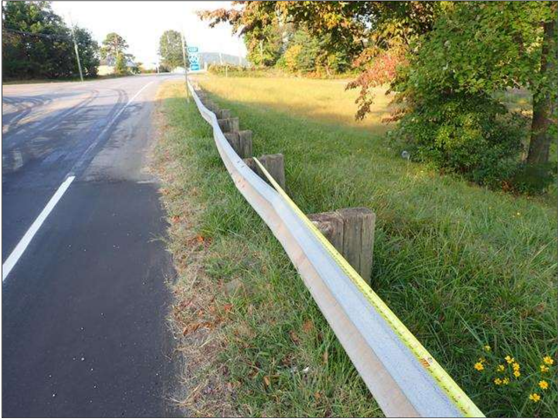
(PAR) southwest guardrail, areas of impact damage (25 feet total)
