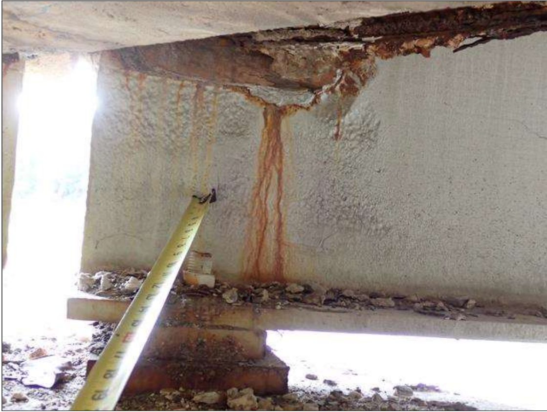
Span 3 Beam 5: (PAR) at bent 3, web adjacent to diaphragm, painted over section loss (5/16 inch average remaining x 4 inch x 6 inch); web over bearing, painted over pitting (up to 1/8 inch deep x 18 inch x 10 inch) with corrosion reinitiated
