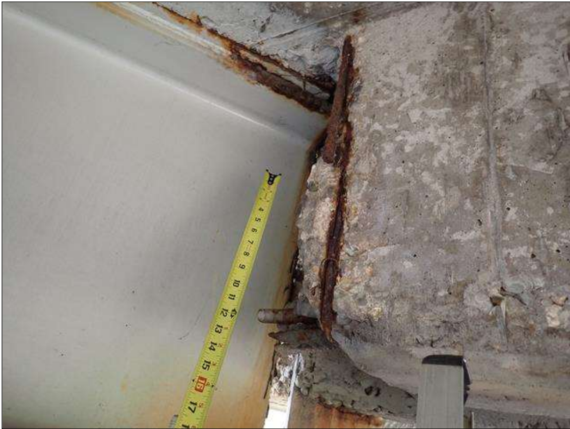
Span 2 Beam 1: end diaphragm on both sides has been removed with exposed rusted rebar, at both ends, when beam was replaced.
