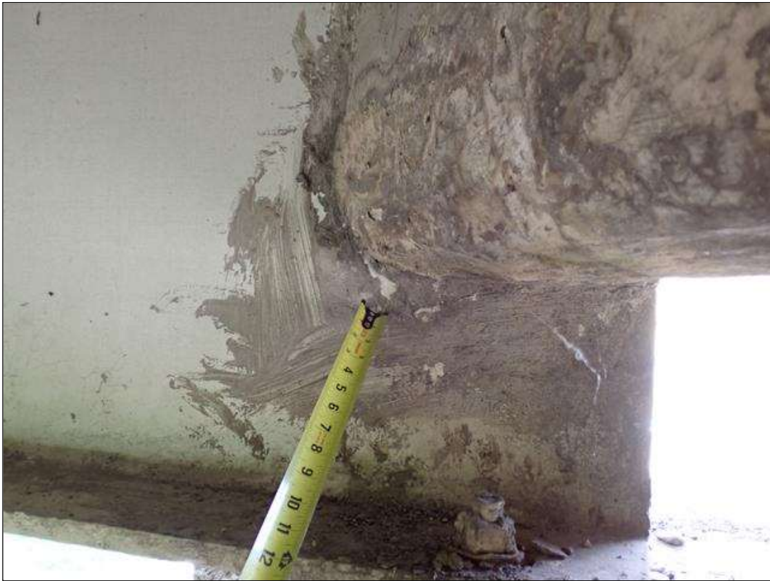
Span 1 Beam 1: (PAR) at bent 1, web adjacent to diaphragm, painted over section loss (3/8 inch average remaining x 9 inch x 2 inch) with corrosion reinitiated
