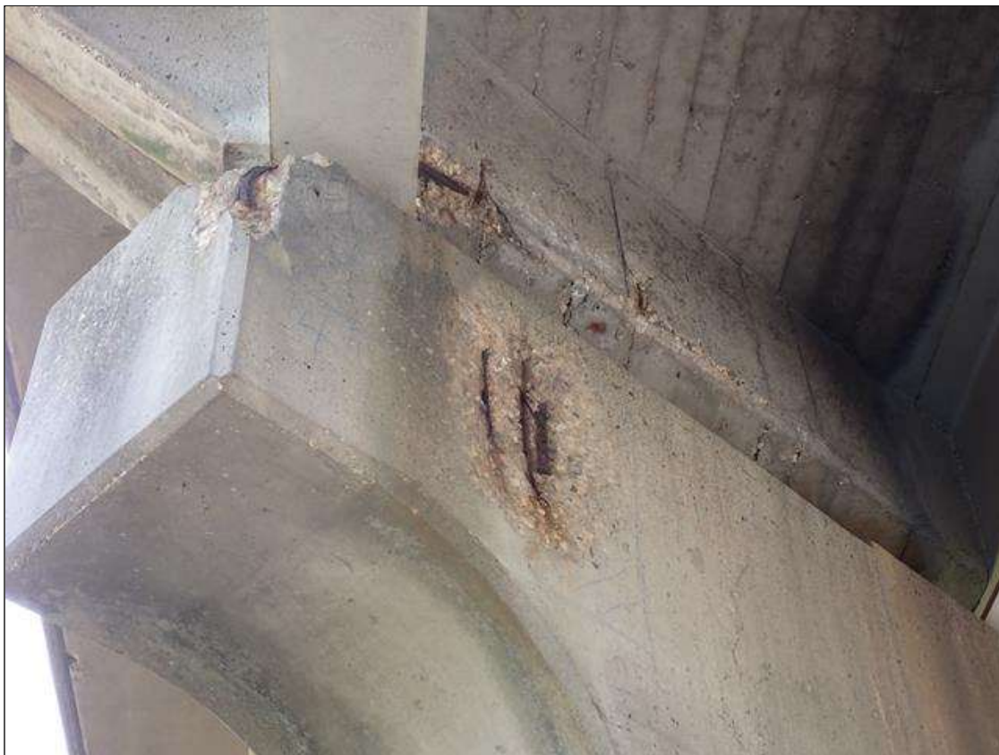
Bent 3 Cap 1: 2 foot x 15 inch x 1 inch deep spall with exposed reinforcing, south face, above column 1
