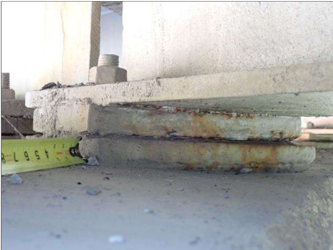
Span 1 Beam 3 - Far Bearing 3: painted over section loss (up to 3/16 inch deep) and pack rust
