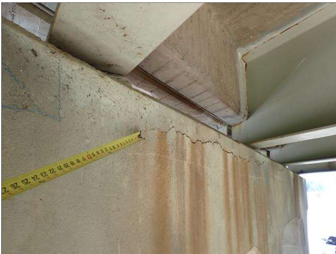
Bent 3 Cap 1: south and north faces, below bays 2-4, delaminations/spalls (up to 10 feet x 2 feet x 1 inch deep) with associated cracks (up to 1/4 inch)
