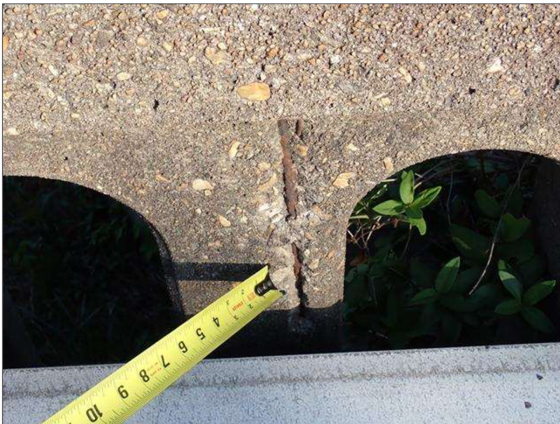
Span 4 Left Bridge Rail: along the length of the rail, spalls (up to 12 inch x 2 inch x 1/2 inch deep) with exposed rusted rebar
