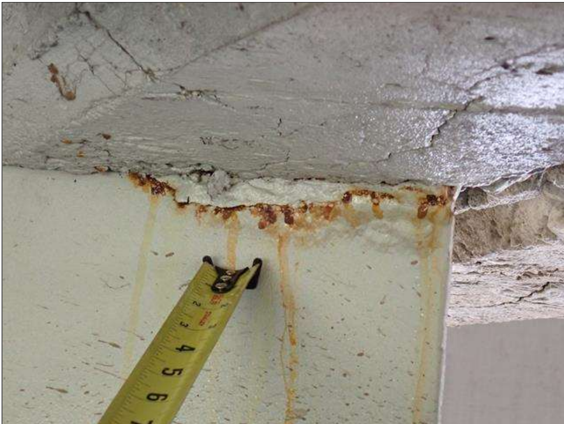
Span 4 Beam 3: (PAR) at bent 3, web adjacent to diaphragm, painted over section loss (3/8 inch average remaining x 8 inch x 1 inch) with corrosion reinitiated
