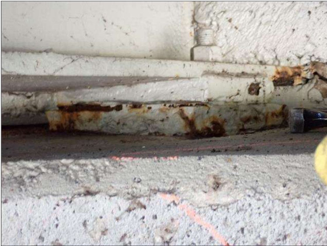
Span 1 Beam 4 - Near Bearing 4: surface rust/rust scale
