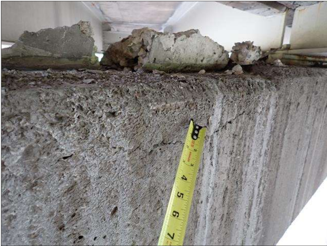
Bent 2 Cap 1: 2.5 foot x 6 inch delamination, with associated cracks up to 1/32 inch wide, south face, under bay 1.
