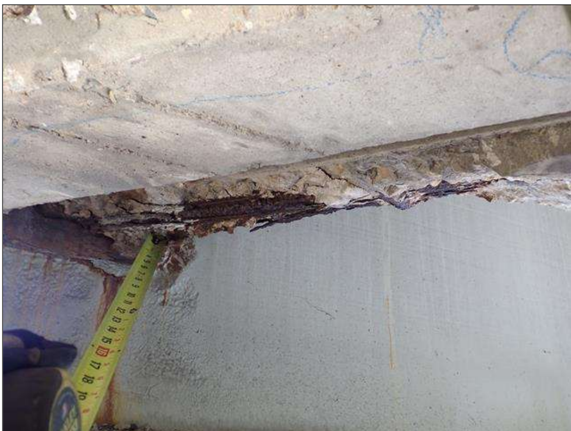
Span 3 Beam 5: 2 - up to 33 inch x 10 inch x 4 inch deep spalls with exposed reinforcing on end diaphragm at both sides of beam, at bents 2 and 3.
