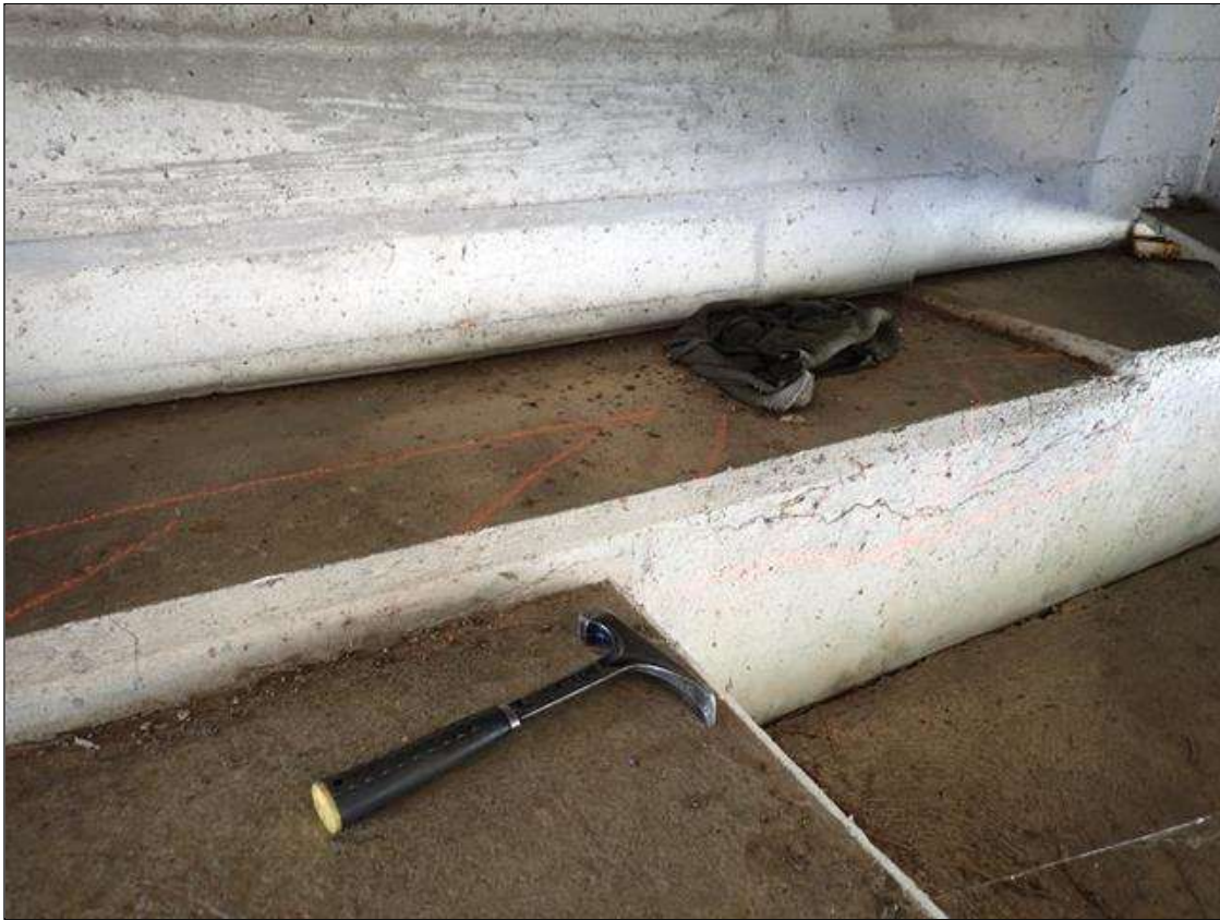
End Bent 1 Cap 1: under bays 3 and 4 on both faces, delaminations [up to 5.5 feet x up to 16 inch] with cracks [up to 1/16 inch]
