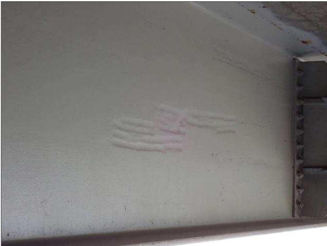
Span 1 Beam 1: inside face of web, previous grinding (up to 1/16 inch deep); areas painted
