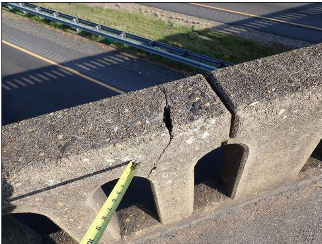
Span 2 Left Bridge Rail: 20 feet from bent 1, diagonal crack (1/8 inch wide) with edge spall (4 inch x 1 inch x 1 inch deep)
