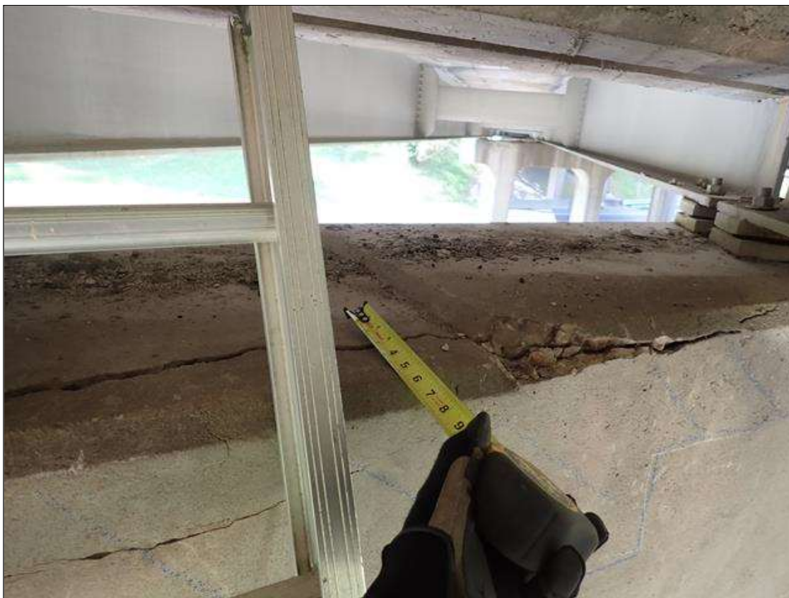
Bent 3 Cap 1: south and north faces, below bays 2-4, delaminations/spalls (up to 10 feet x 2 feet x 1 inch deep) with associated cracks (up to 1/4 inch)
