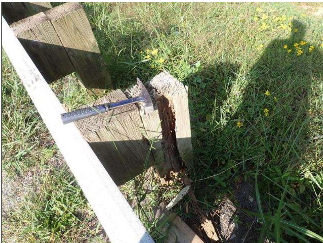
(PAR) southwest guardrail transition, (1) decayed post
