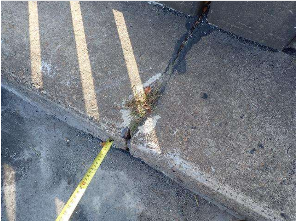
Span 2 Expansion Joint at Bent 1: both sidewalks, seal damaged/missing
