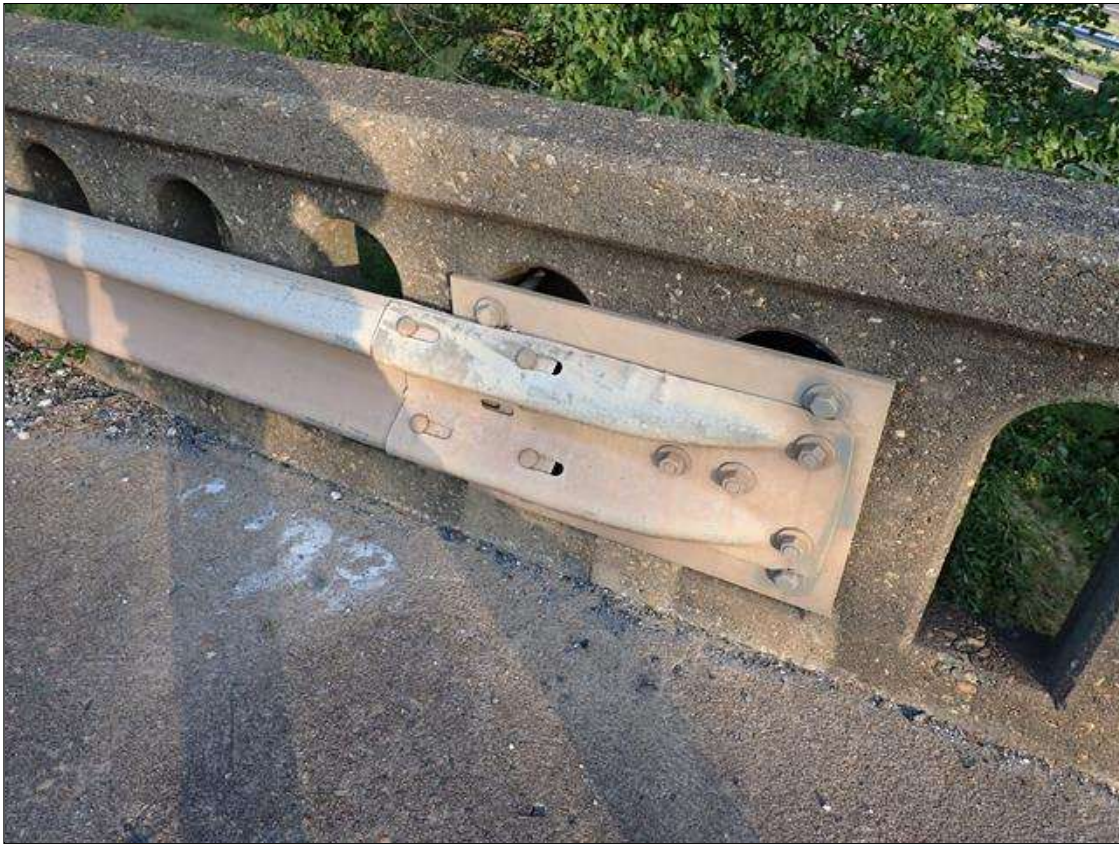
southwest guardrail attachment
