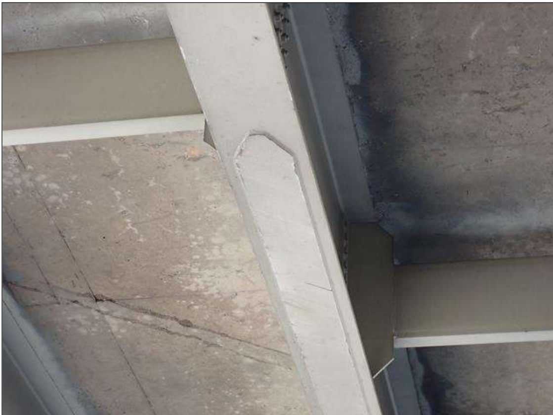
Span 3 Beam 3: over right travel lane, along bottom flange at cover plate, impact scrapes with surface gouges
