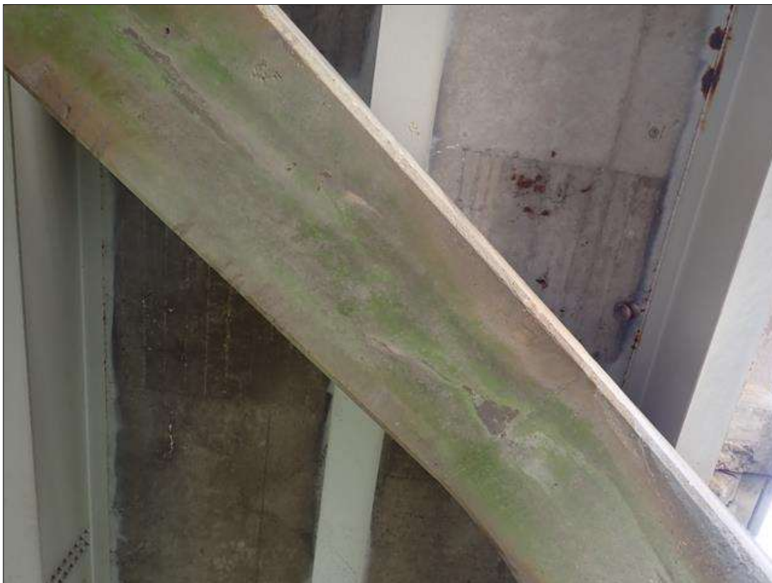
Bent 1 Cap 1: (not found 2023) 2 foot transverse crack up to 1/32 inch wide, under beam 2, on underside of cap.
