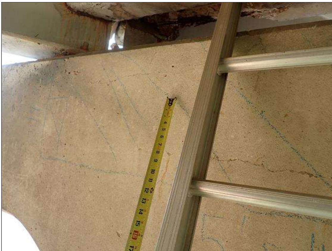
Bent 3 Cap 1: south and north faces, below bays 2-4, delaminations/spalls (up to 10 feet x 2 feet x 1 inch deep) with associated cracks (up to 1/4 inch)
