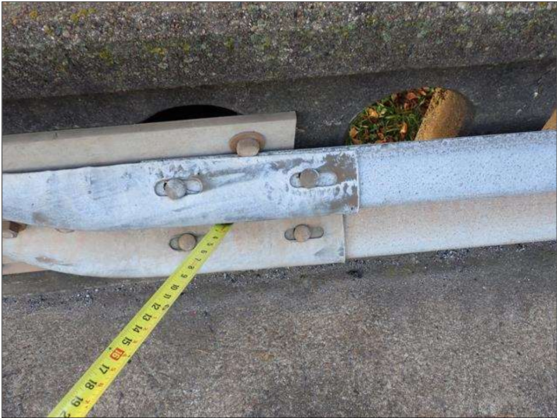
(PAR) southeast guardrail attachment, improper lap
