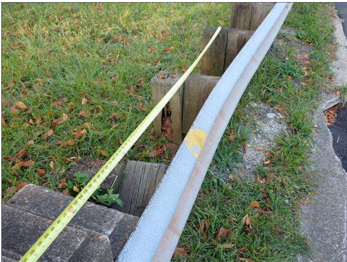
(PAR) southeast guardrail transition, impact damage (7 feet) with (1) decayed post
