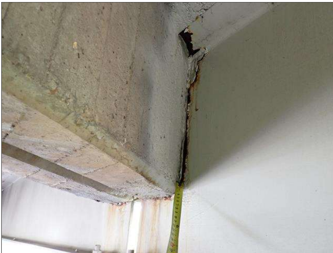
Span 1 Beam 5: (PAR) at bent 1, web adjacent to diaphragm, painted over section loss (5/16 inch average remaining x 9 inch x up to 2 feet) with corrosion reinitiated; top flange, rust scale
