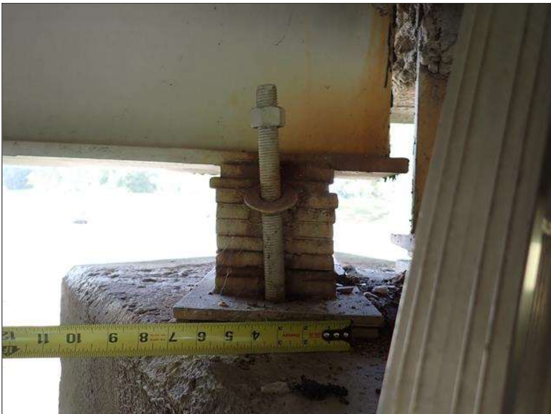
Span 2 Beam 1 - Far Bearing 1: (PAR) stacked plates, laterally misaligned (up to 1/2 inch) in relation to sole plate; no anchor bolts installed through beam and masonry plate anchor bolts too long with disengaged nuts
