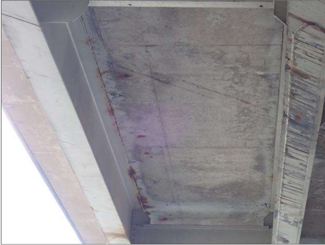
Span 2 Deck: (PAR) throughout underside of deck, in all bays, transverse cracks (up to 1/32 inch x full width) and areas of map cracks (hairline) with efflorescence buildup and some rust stains
