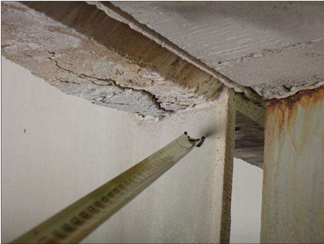
Span 3 Beam 3: (PAR) at bent 3, web adjacent to diaphragm, painted over section loss (5/16 inch average remaining x 10 inch x 1 inch)
