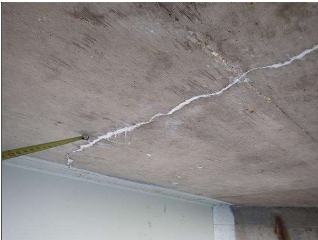
Span 1 Deck: (PAR) underside of all bays, transverse and map cracks (up to 1/32 inch) with efflorescence buildup and some rust stains at random
