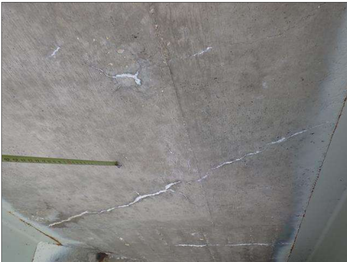
Span 4 Deck: (PAR) underside of all bays, near bent 3 and end bent 2, transverse cracks (up to 1/32 inch x full width) and map cracks (hairline) with efflorescence buildup and some rust stains at random
