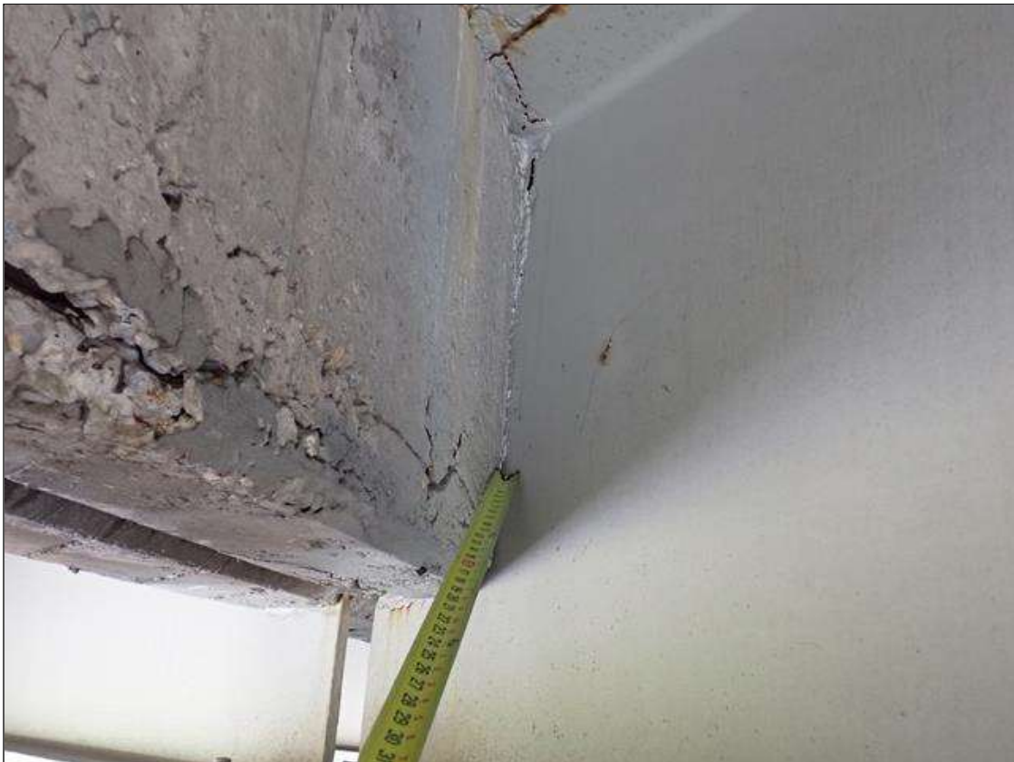
Span 2 Beam 2: at bent 2, web adjacent to diaphragm, painted over section loss (7/16 inch average remaining x 4 inch x 1 inch) with corrosion reinitiated; top flange, upper web and bottom flange, rust scale
