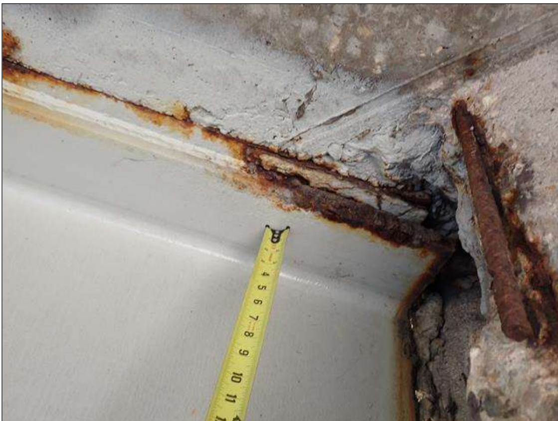
Span 2 Beam 1: at bent 2, top flange, rust scale
