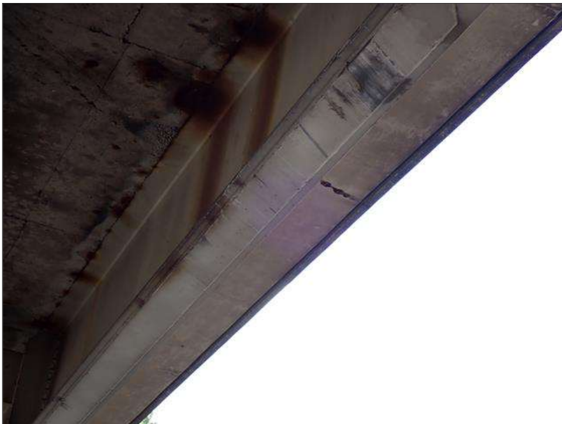
Span 3 Beam 1: over both travel lanes, along underside of cover plate, impact scrapes with surface gouges
