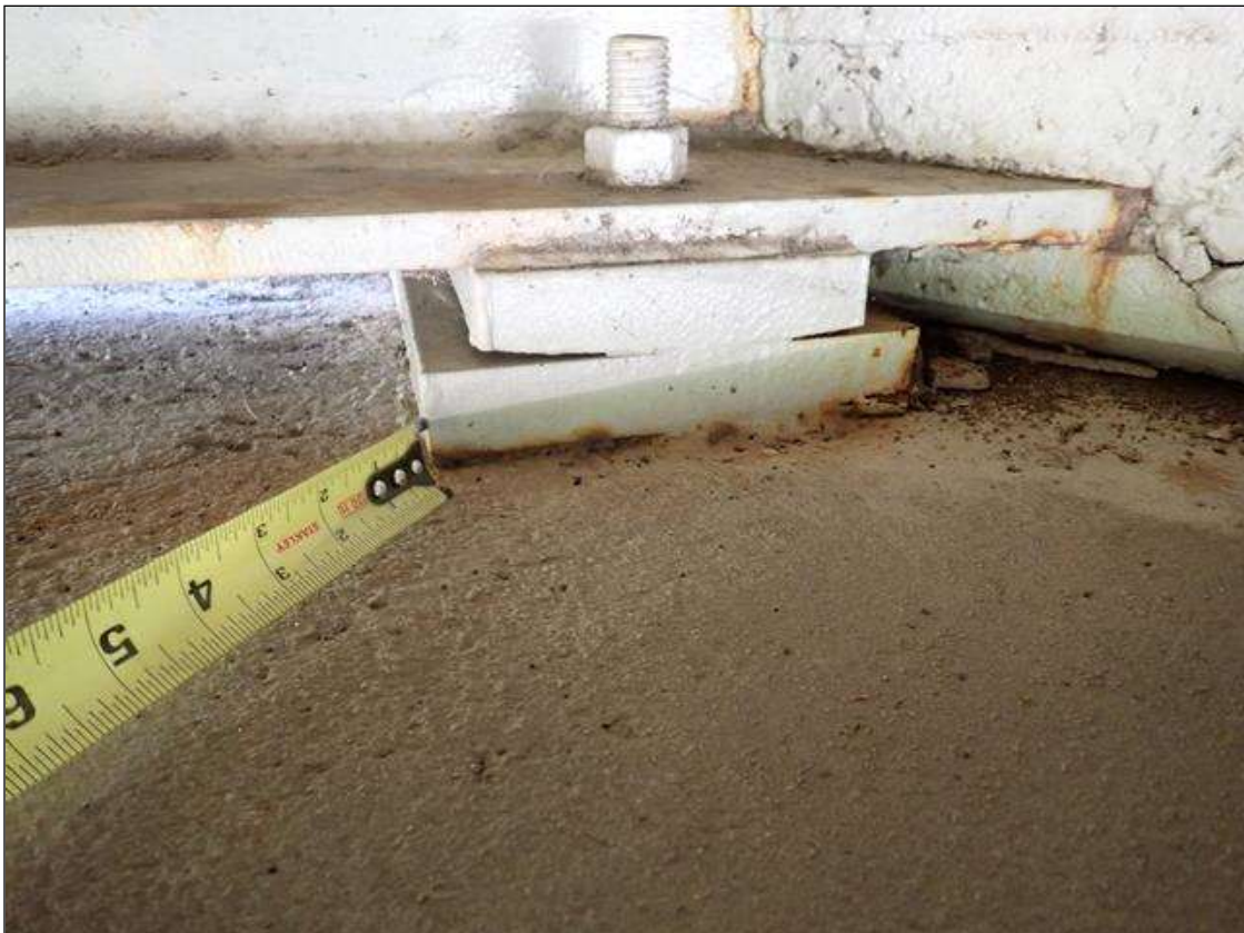
Span 4 Beam 1 - Far Bearing 1: freckled rust
