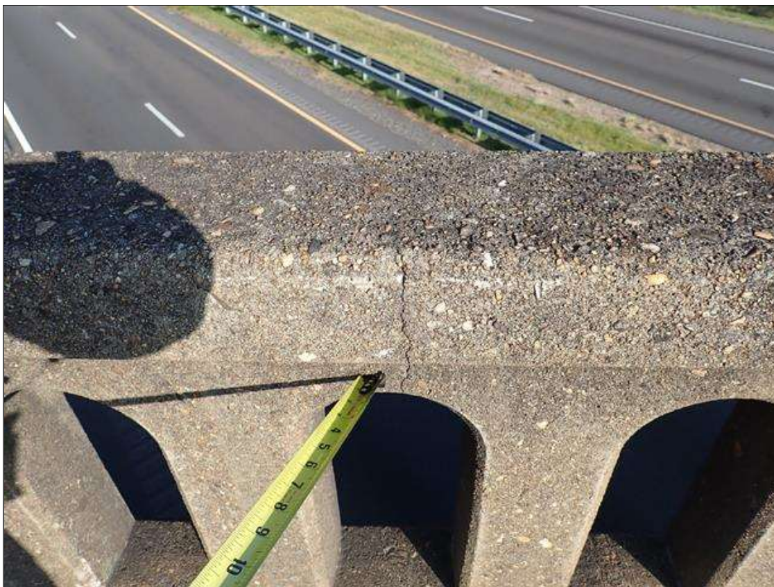
Span 2 Left Bridge Rail: near bent 1, vertical cracks (up to 1/32 inch x 9 inches)
