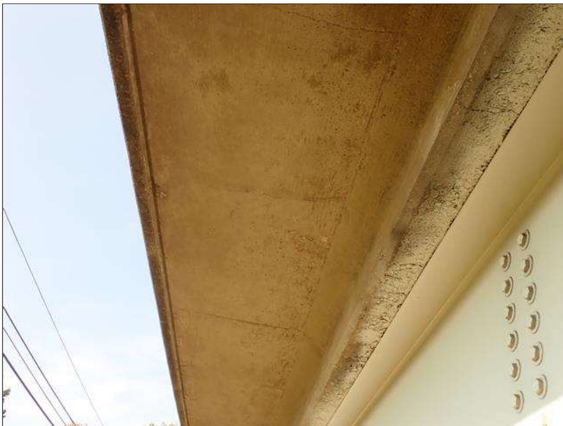
Span 4 Deck: underside of both overhangs, transverse cracks up to 1/32 inch wide x full width, intermittent length of span
