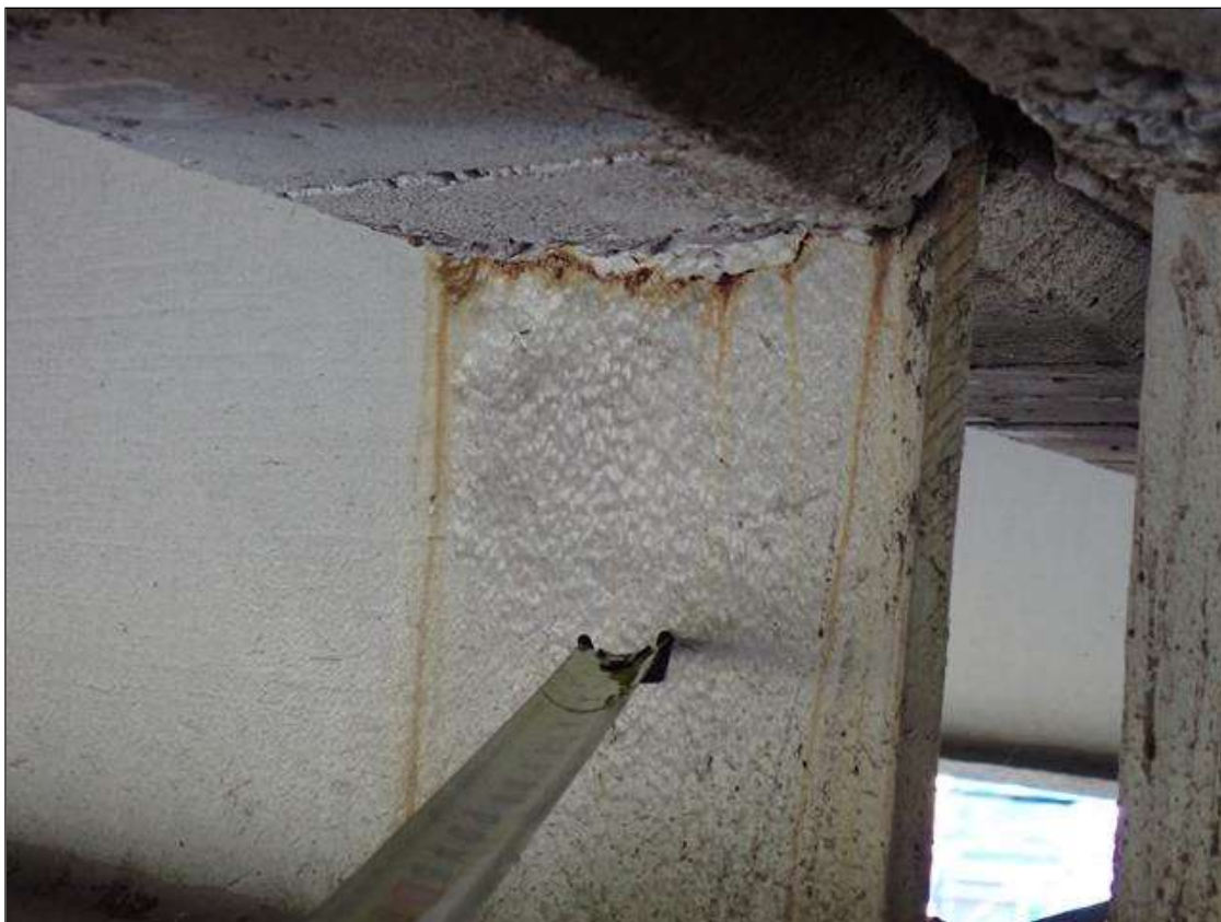
Span 3 Beam 4: (PAR) at bent 2, web adjacent to diaphragm, painted over section loss (3/8 inch average remaining x 9 inch x 5 inch) with corrosion reinitiated
