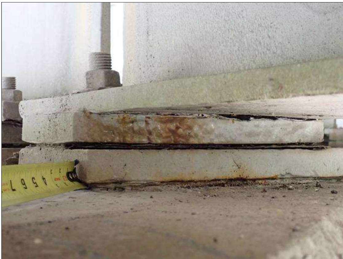
Span 4 Beam 4 - Near Bearing 4: painted over section loss (up to 1/8 inch deep) and pack rust
