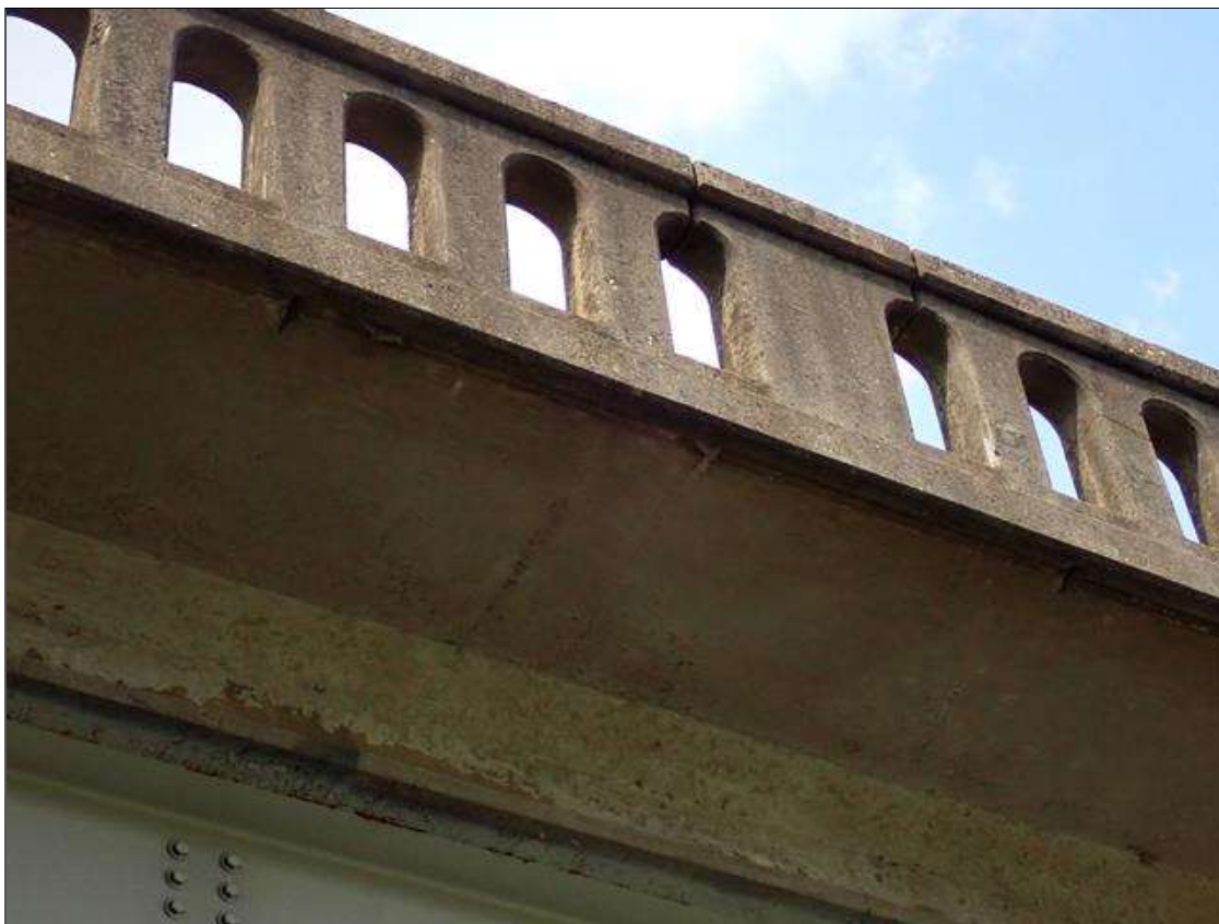
Span 2 Deck: (PAR) 8 - spalls with exposed reinforcing up to 2 inch diameter x 1/2 inch deep, underside of right overhang, at random.
