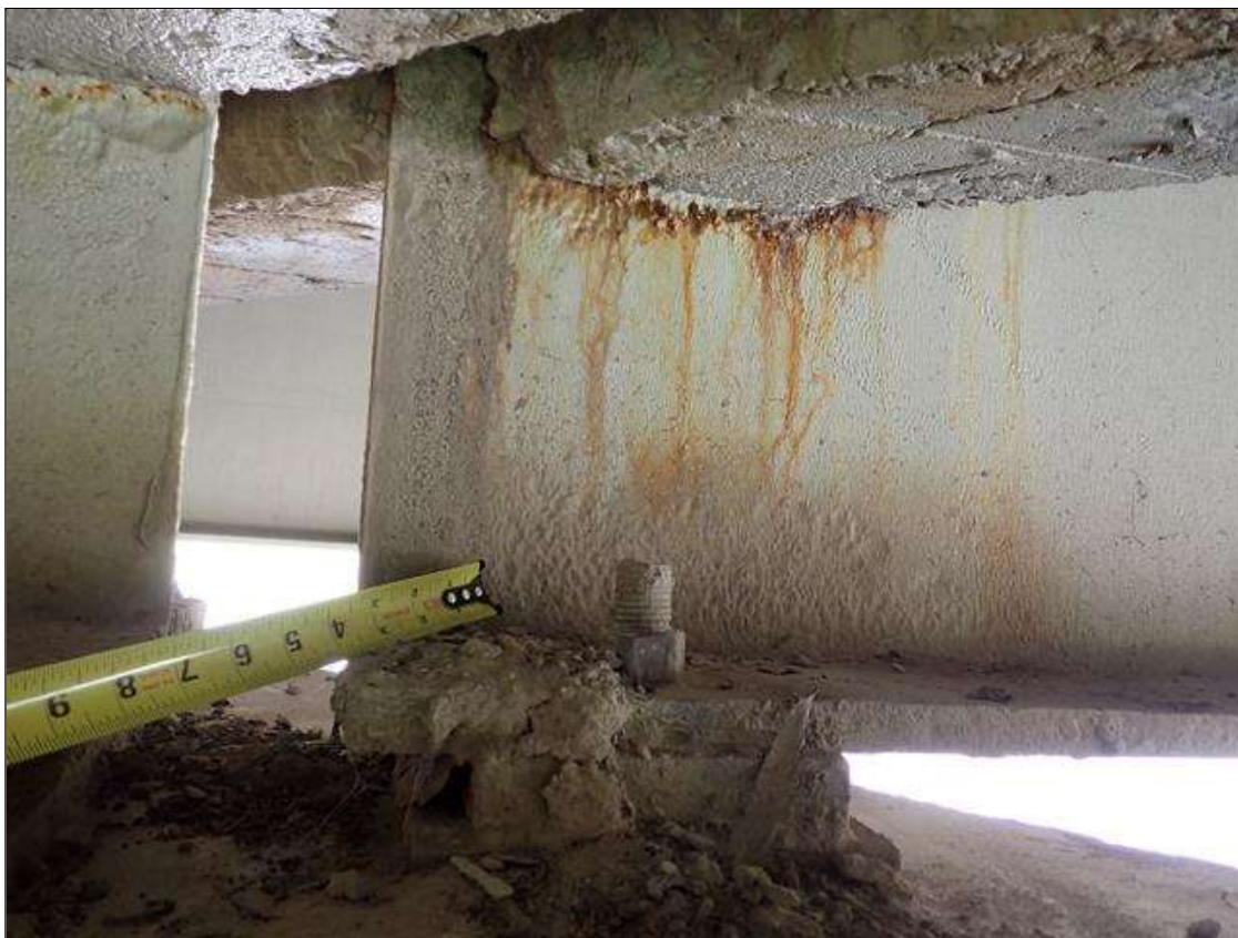
Span 2 Beam 3: (PAR) at bent 1, web adjacent to diaphragm, painted over section loss (5/16 inch average remaining x 6 inch x 1 inch); lower web, painted over pitting (up to 1/8 inch deep x 14 inch x 3 inch) with corrosion reinitiated
