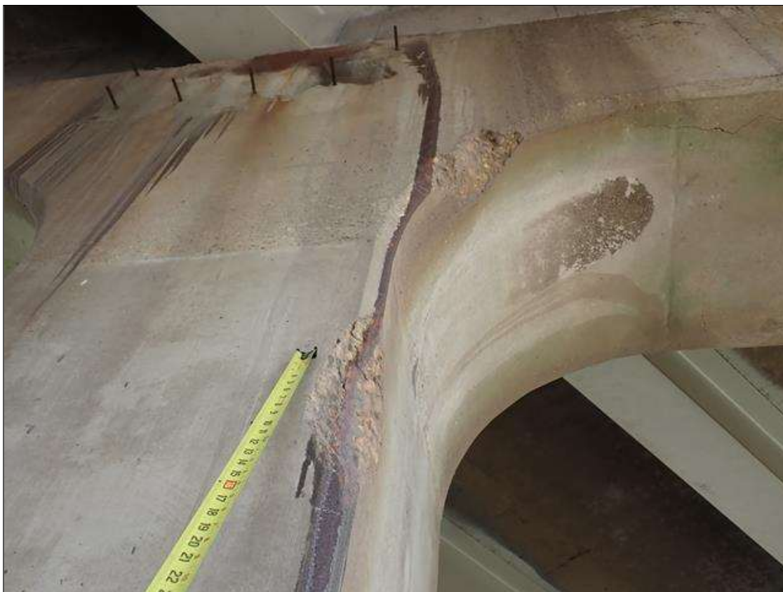
Bent 2 Pile 2: 2 - spalls up to 15 inch x 6 inch x 1.5 inch deep [no exposed rusted reinforcing] south face, at corbel near top of column.
