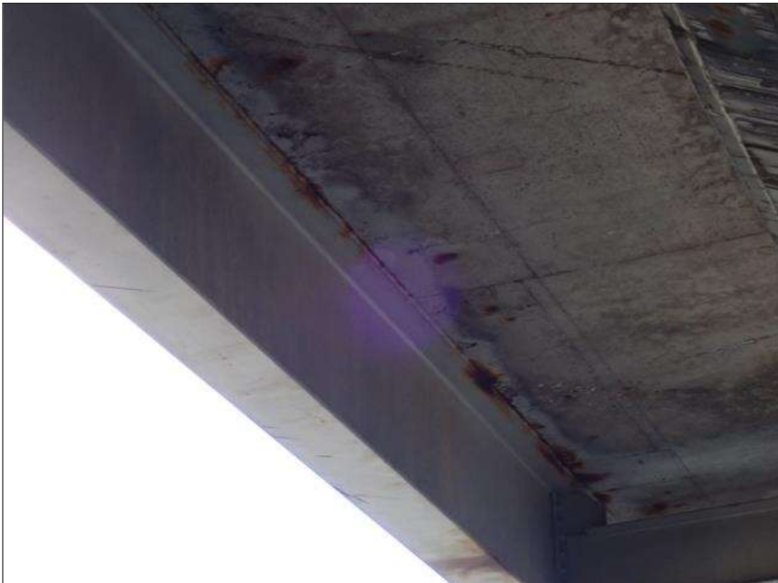
Span 2 Beam 1: surface rust at edges of top and bottom flange, at random, along beam.
