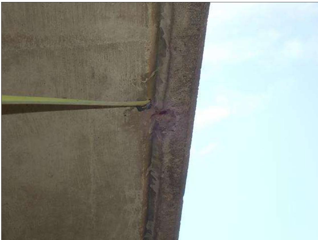
Span 4 Deck: (PAR) 3 - spalls with exposed reinforcing up to 1 inch diameter x 1/2 inch deep, underside of left overhang, intermittent length of span.
