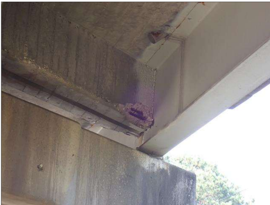
Span 4 Beam 1: at bent 3, bay 1 end diaphragm, spall (2 feet x 10 inch x 2 inch deep) with exposed rusted rebar
