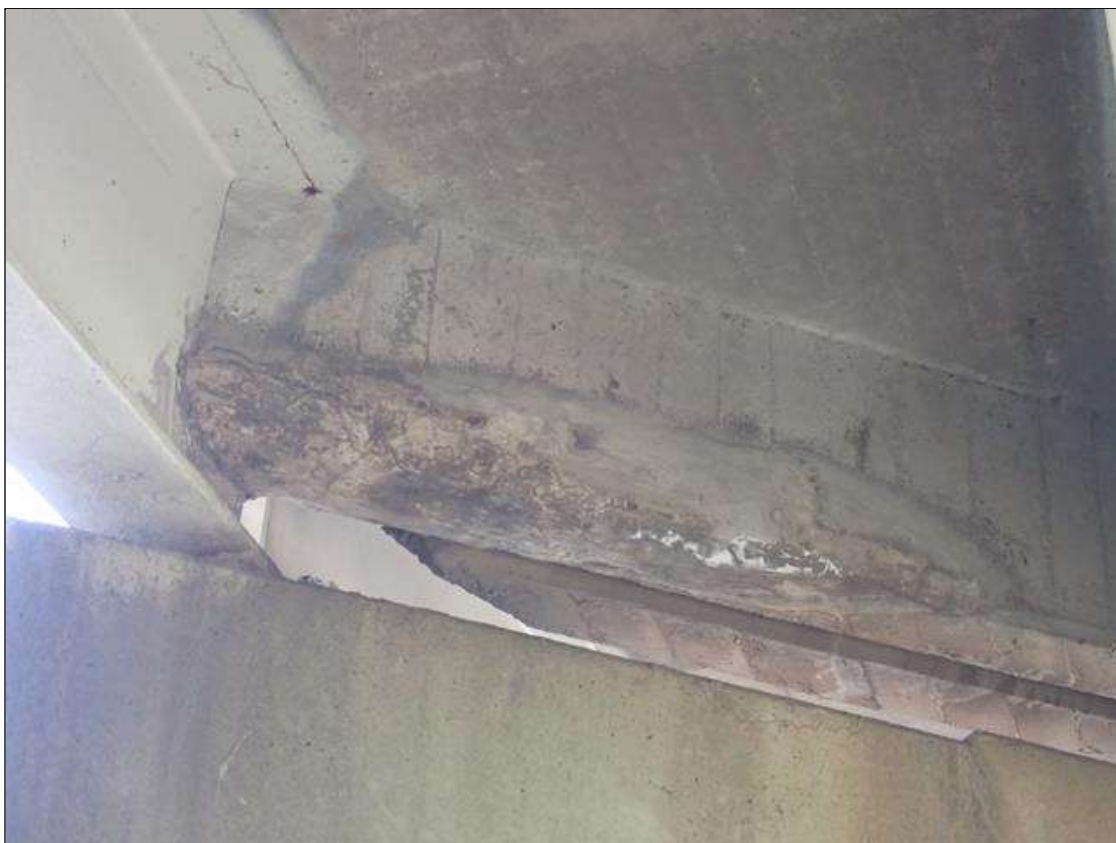
Span 1 Beam 1: bent 1 end diaphragm at bent 1, patched area (4.5 foot x 1 foot) with hairline cracks with efflorescence; adjacent to beam 2, delamination (1 foot x 6 inch)
