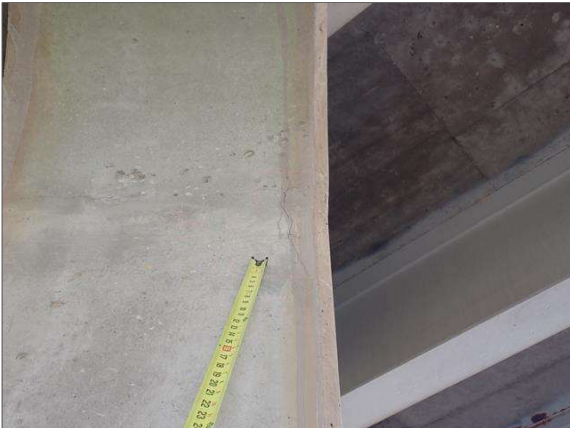
Bent 1 Pile 2: at Northeast corner adjacent to corbel, delamination [8 inch x 13 inch]
