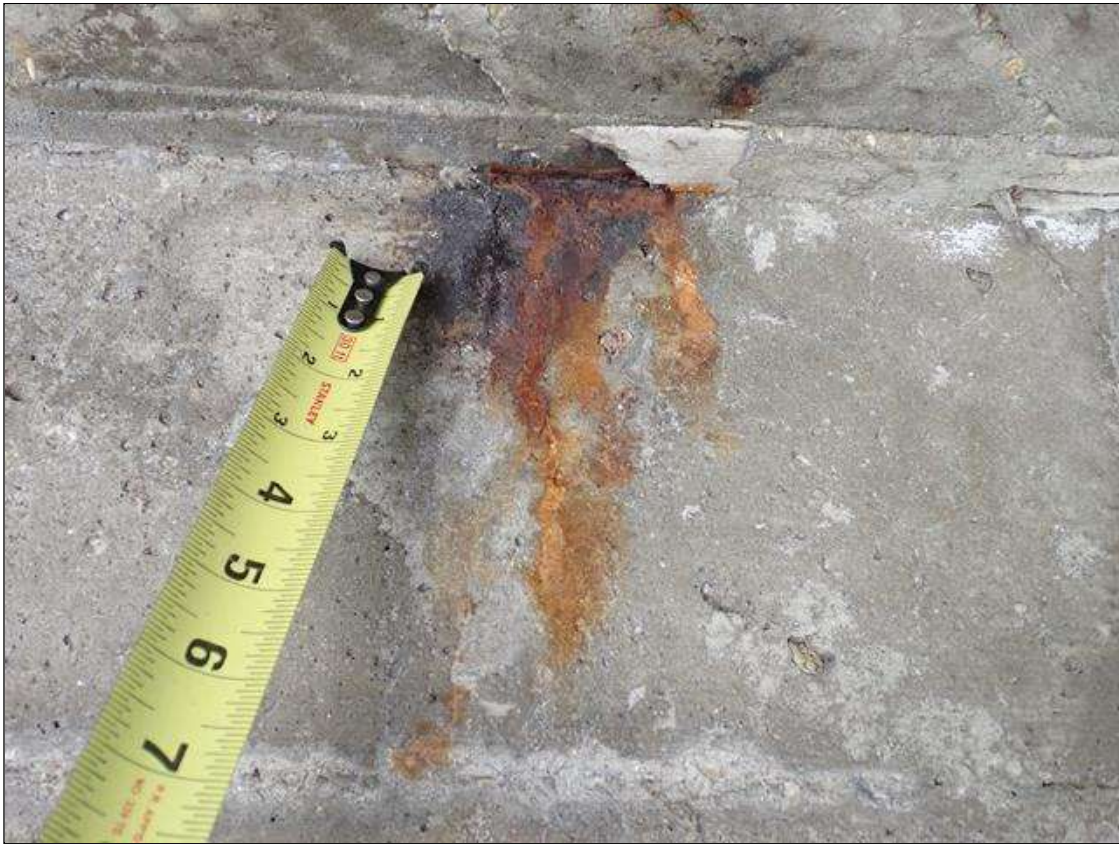
End Bent 2 Abutment: (PAR) top of abutment, in bay 3, rust stains
