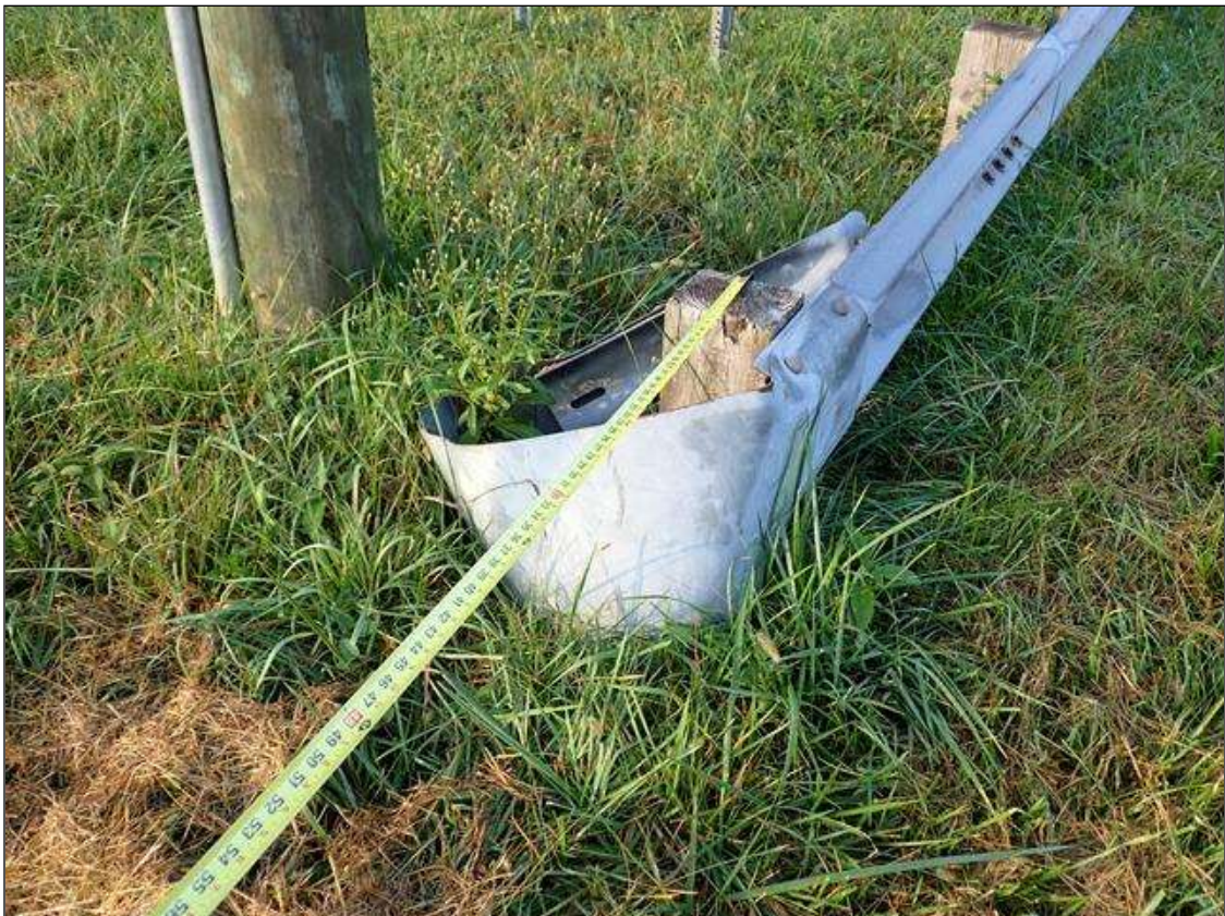
(PAR) northeast guardrail termination, impact damage (1 foot)
