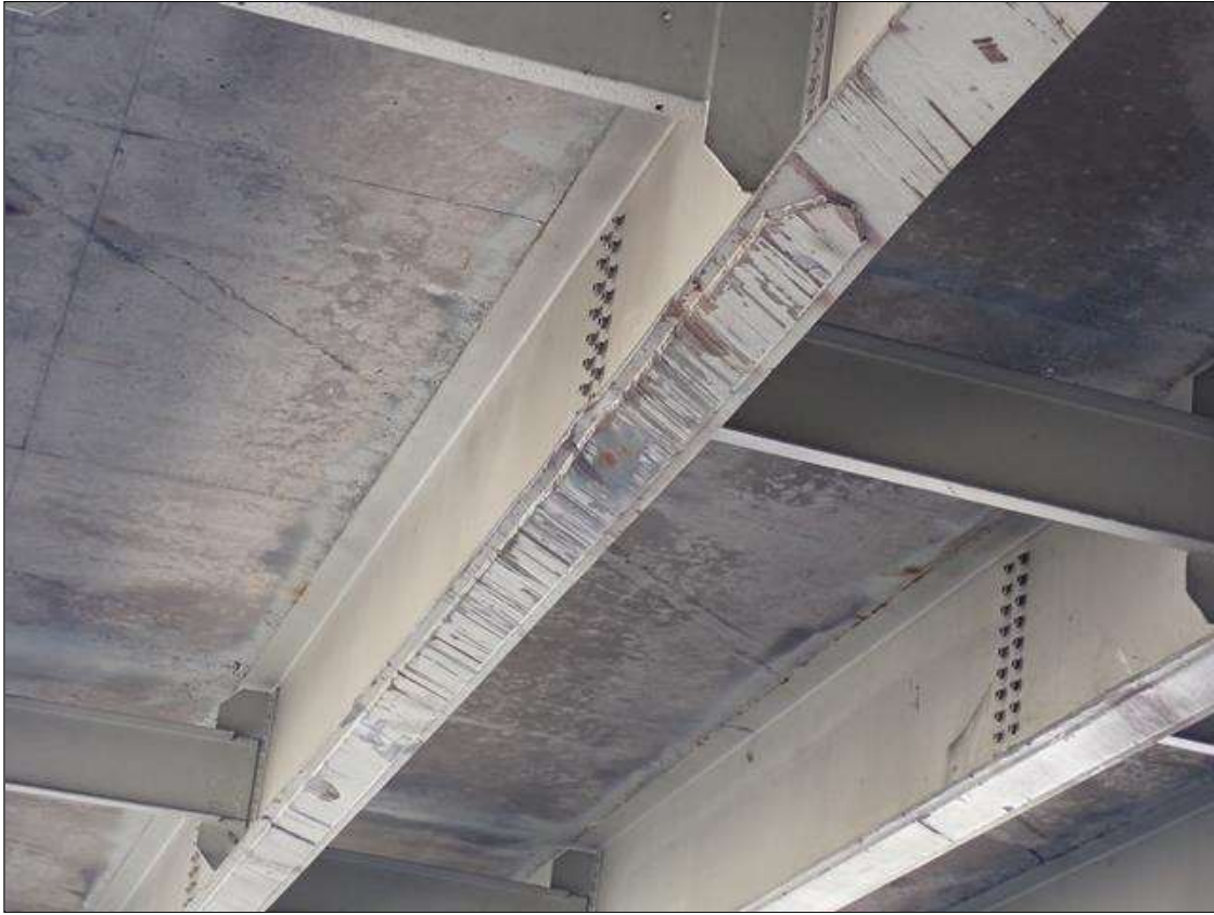
Span 2 Beam 2: (PAR) over both travel lanes, underside of bottom flange and cover plate, impact scrapes with gouges (up to 1/2 inch deep); over right travel lane, bottom flange and cover plate, distorted (up to 1 inch upwards x approximately 1.5 feet); no apparent distress to cover plate welds
