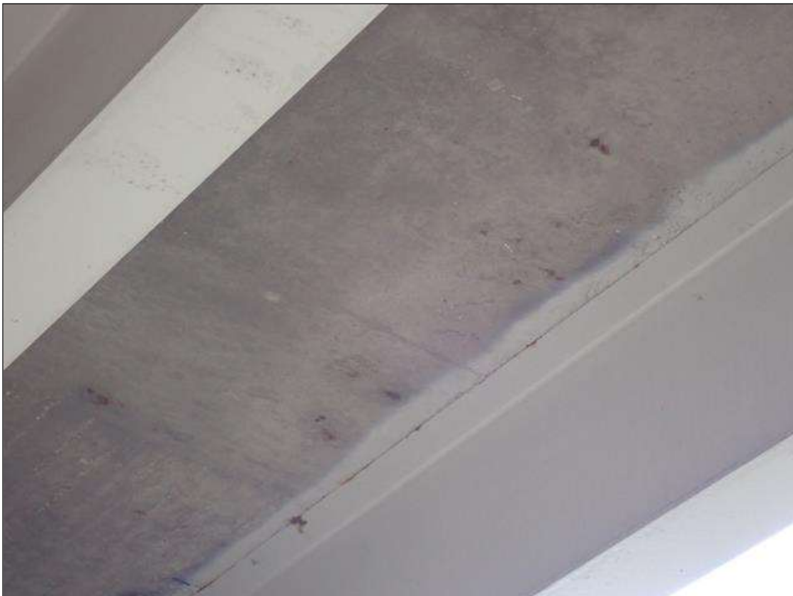
Span 4 Deck: (PAR) underside of all bays, near bent 3 and end bent 2, transverse cracks (up to 1/32 inch x full width) and map cracks (hairline) with efflorescence buildup and some rust stains at random
