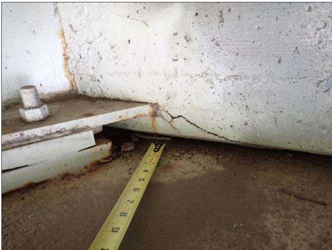
End Bent 2 Abutment: delamination up to 6 inch x 8 inch, east side of beam 3 (typical at all beams at end bent 2).
