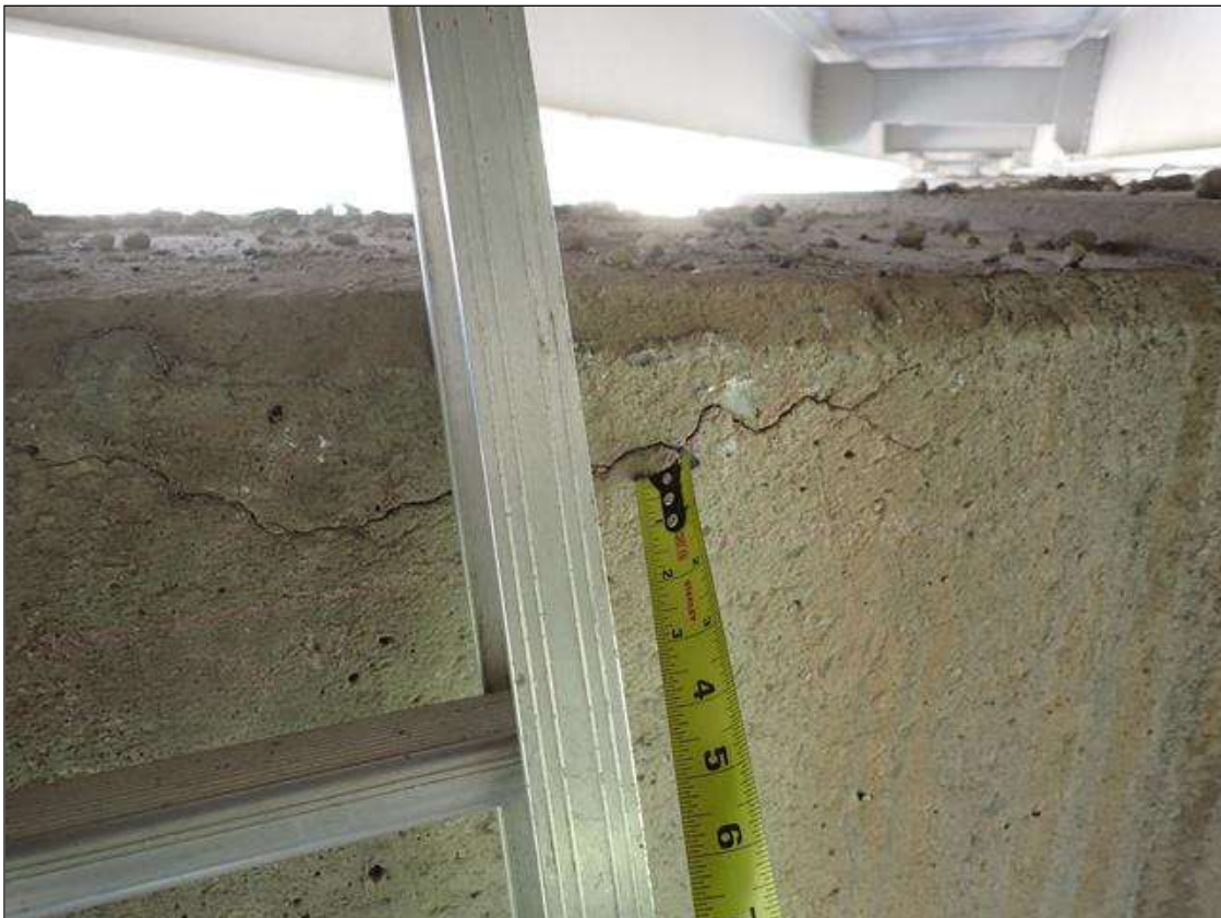
Bent 1 Cap 1: south face, below bay 1, longitudinal crack (1/32 inch x 15 inches)
