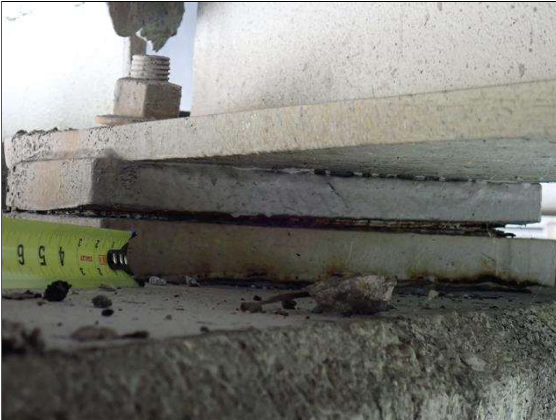
Span 1 Beam 2 - Far Bearing 2: pack rust.
