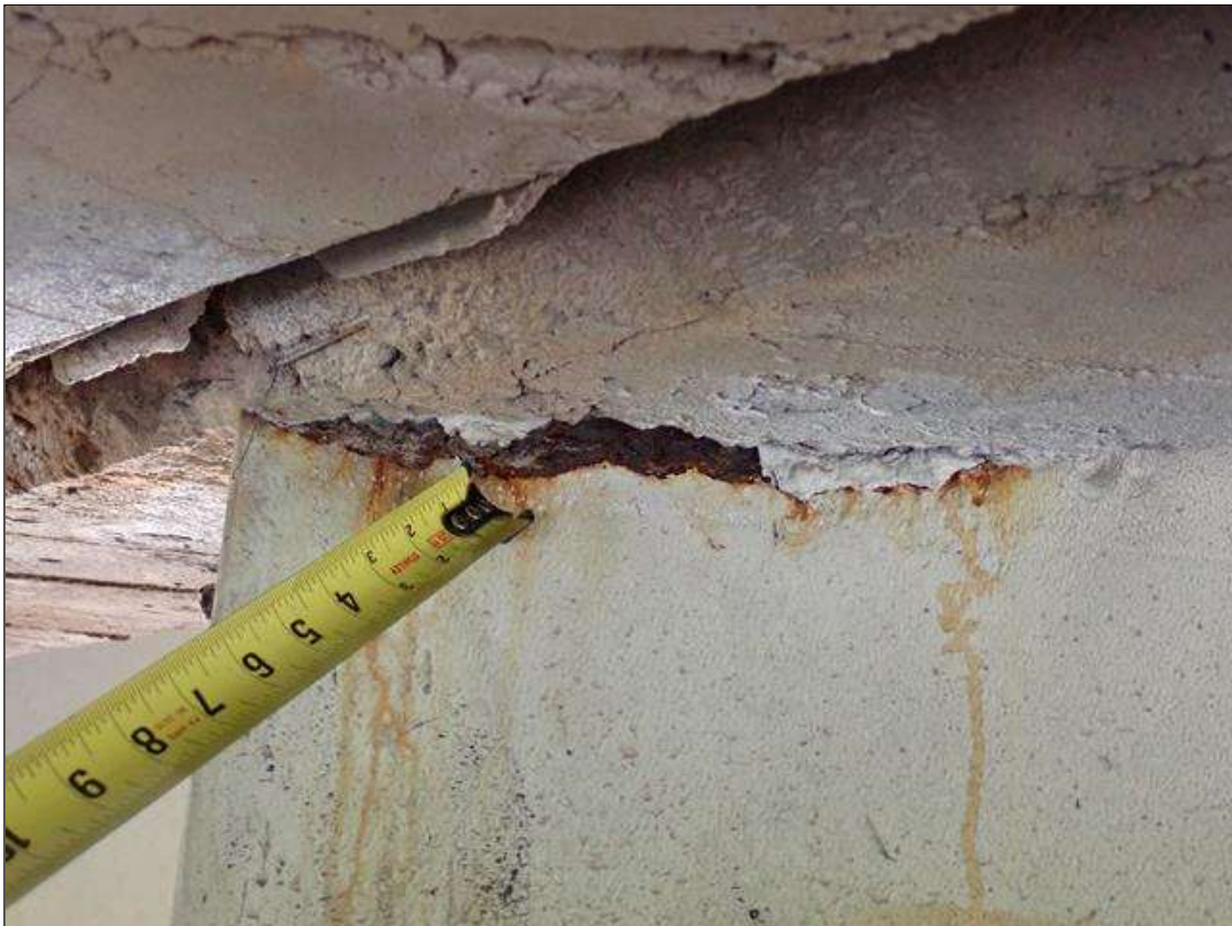
Span 3 Beam 3: (PAR) at bent 2, web adjacent to diaphragm, painted over section loss (3/8 inch average remaining x 10 inch x 1 inch) with corrosion reinitiated
