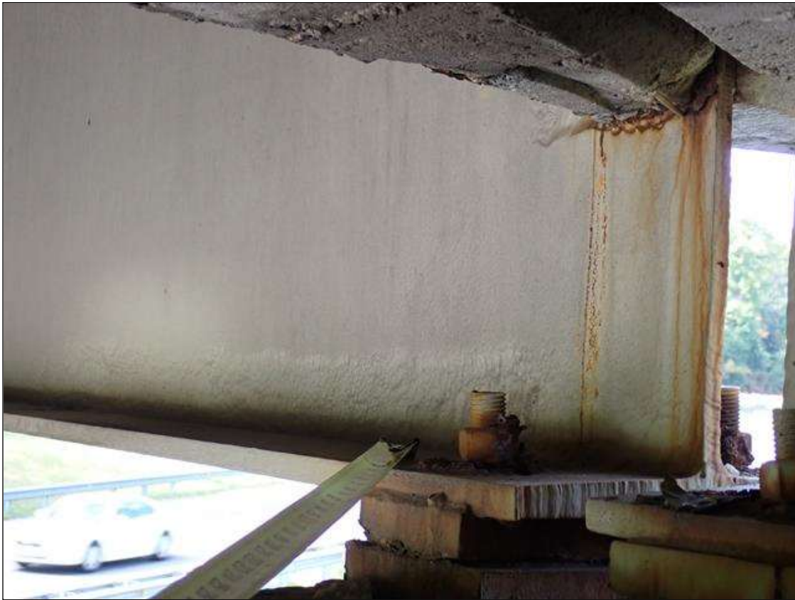
Span 3 Beam 1: (PAR) at bent 3, painted over section loss: web adjacent to diaphragm (5/16 inch average remaining x 9 inch x 2 inch); lower web (3/8 inch average remaining x 4 feet x 4 inch) with corrosion reinitiated
