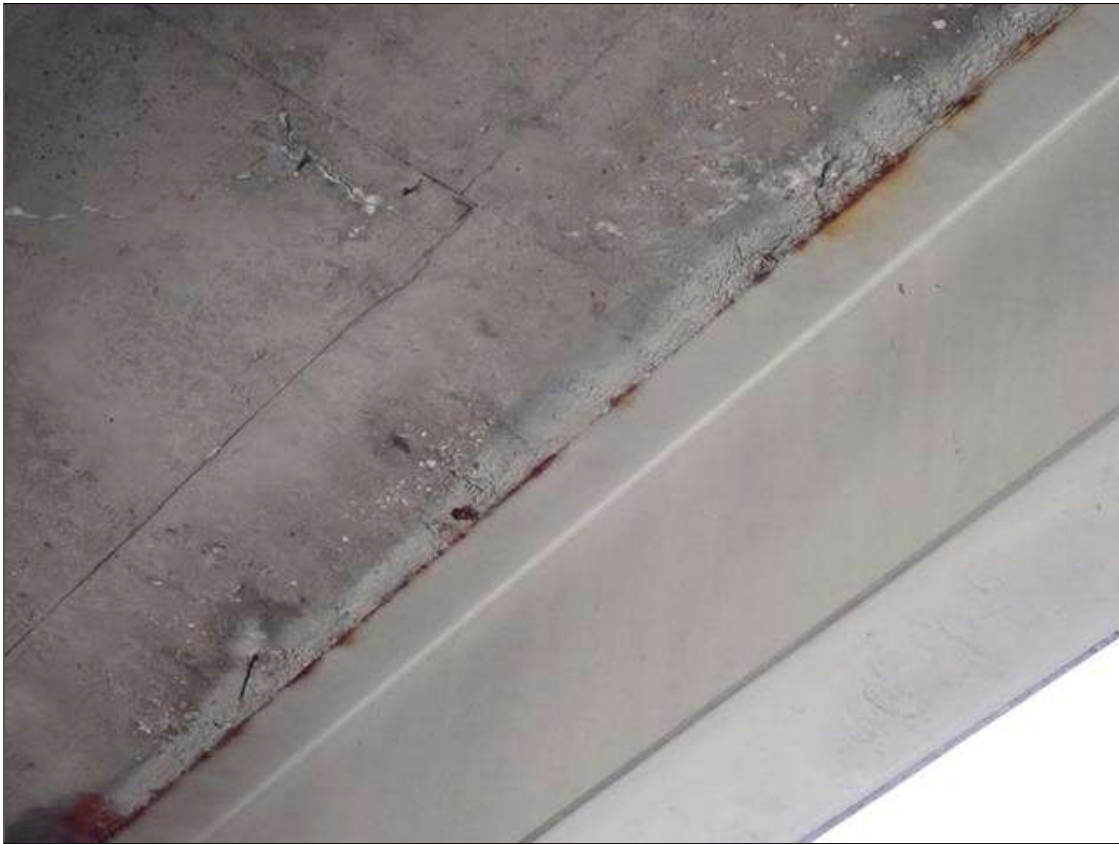
Span 3 Beam 1: along the length of the beam, along edges of top flange, surface rust at random
