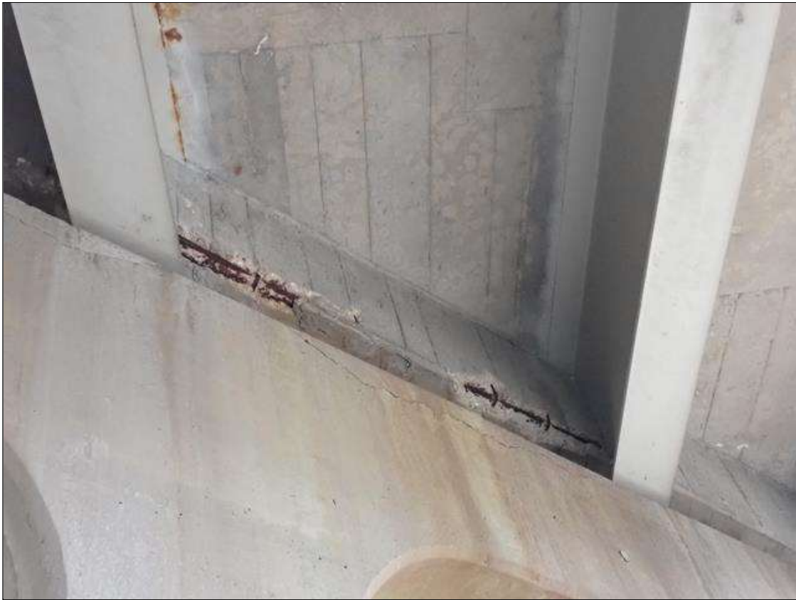
Span 3 Beam 3: at bent 3, bay 3 end diaphragm, spalls (up to 3 feet x 6 inch x 2 inch deep) with exposed rusted rebar
