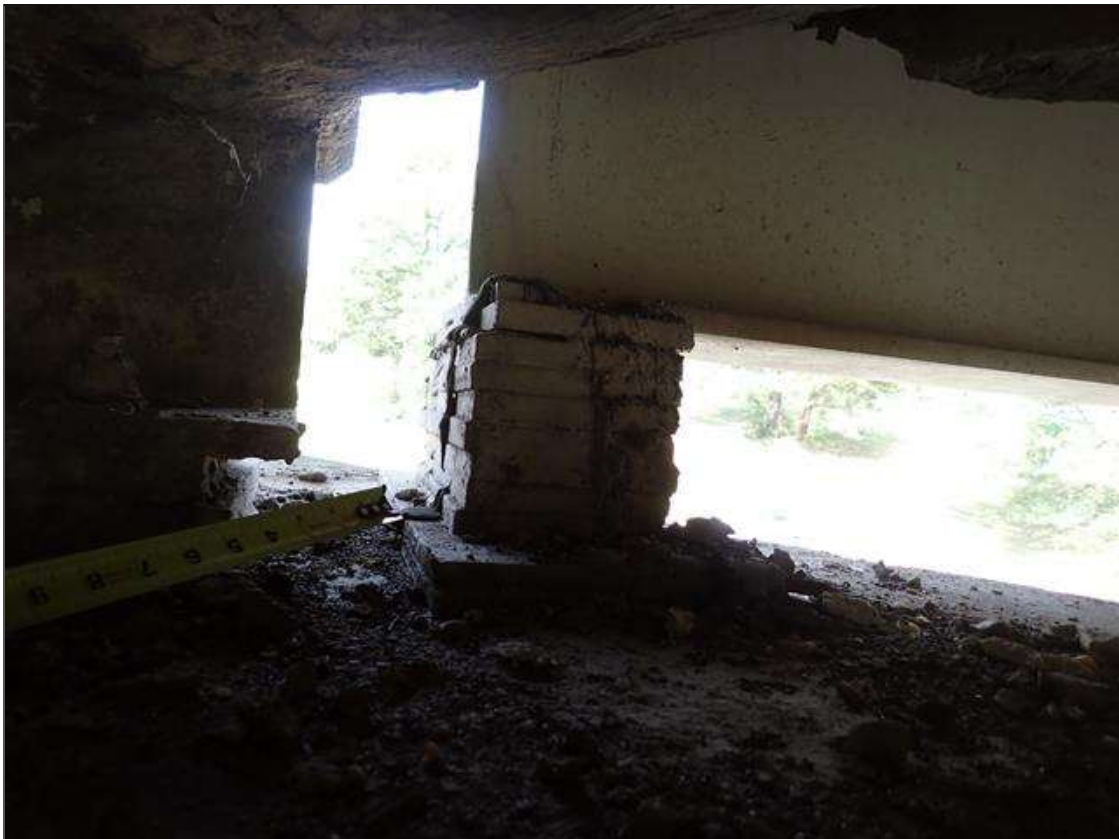
Span 2 Beam 1 - Near Bearing 1: (PAR) stacked plates, laterally misaligned (up to 1/2 inch) in relation to sole plate; no anchor bolts installed through beam or into cap
