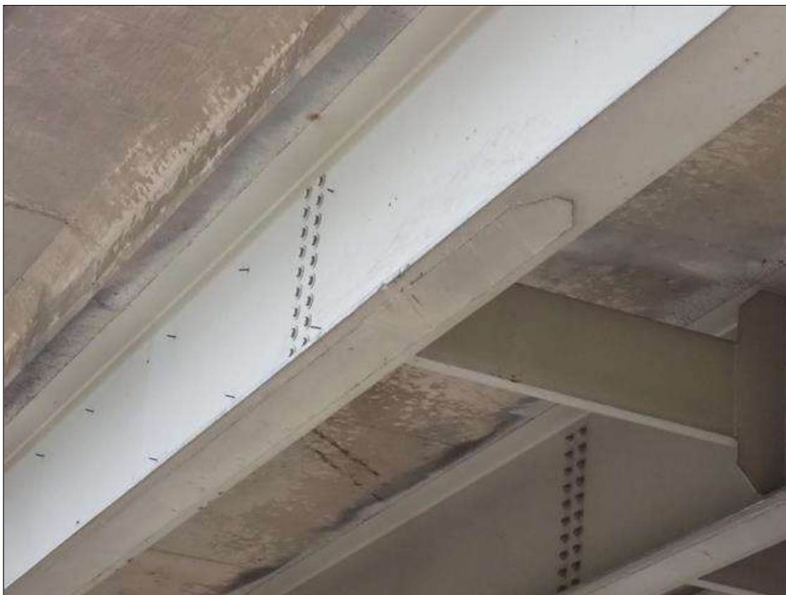
Span 3 Beam 5: over right travel lane, along underside of bottom flange and cover plate, impact scrapes and gouges (approximately 1/2 inch deep)
