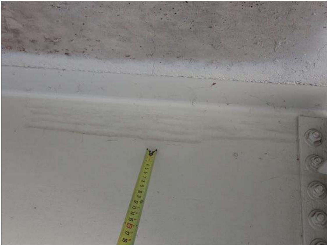
Span 1 Beam 1: inside face of web, previous grinding (up to 1/16 inch deep); areas painted
