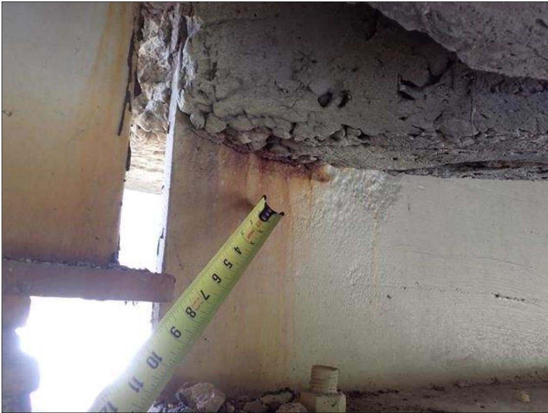
Span 3 Beam 1: (PAR) at bent 2, web adjacent to diaphragm, painted over section loss (3/8 inch average remaining x 14 inch x 4 inch) with corrosion reinitiated
