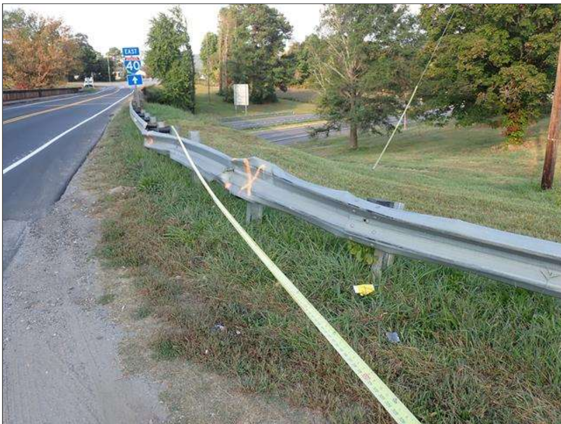
(PAR) northwest guardrail, impact damage (38 feet)
