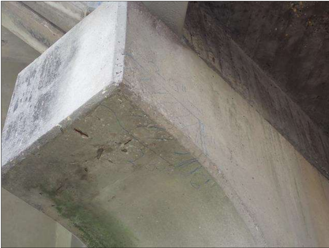
Bent 1 Cap 1: at Northeast corner, lower edge, delamination [20 inch x 1 foot]
