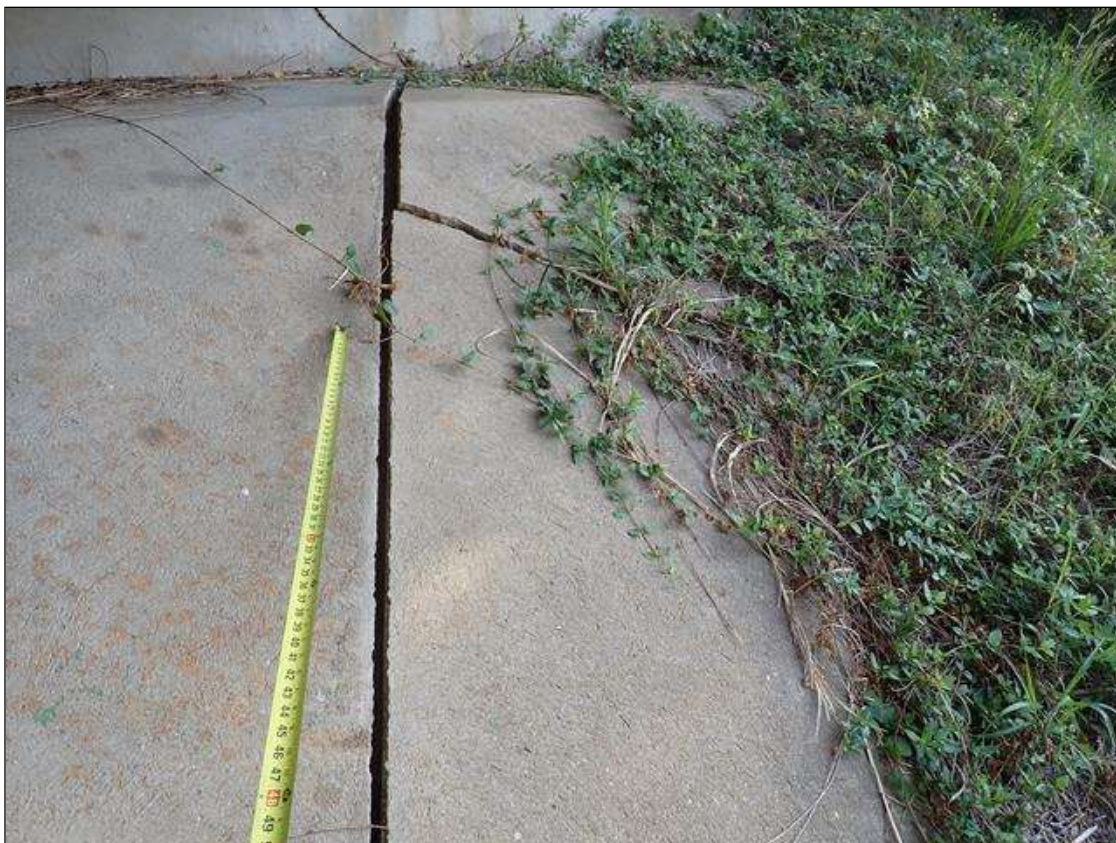
end bent 2 slope protection, at east end, section settled/shifted to the east (up to 1.5 inch) with adjacent transverse crack (up to 1 inch wide x 6 feet)
