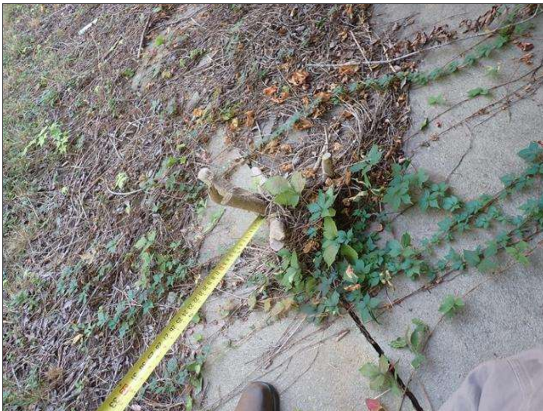
end bent 1 slope protection, west end, tree growing between sections; section settled/shifted to the west (up to 1 inch)
