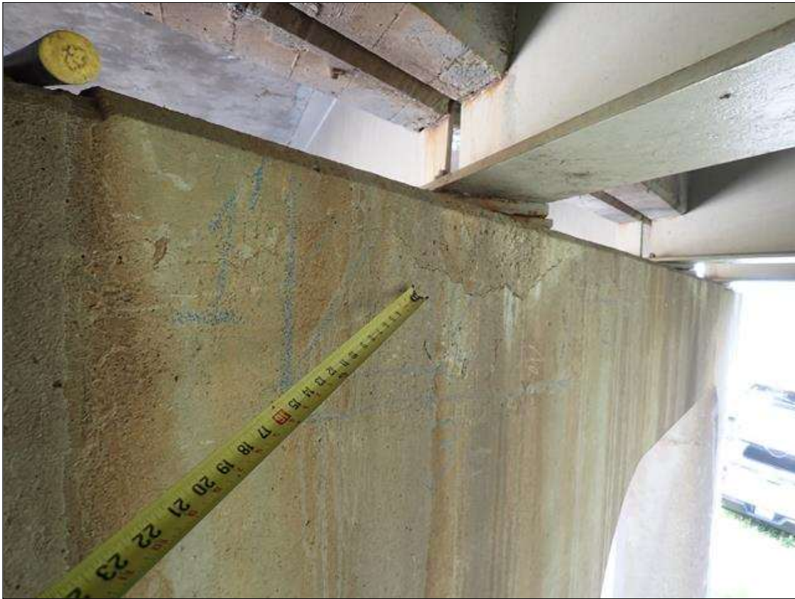
Bent 1 Cap 1: south face, below beam 3, delamination (6 feet x 1 foot) with associated cracks (up to 1/32 inch)
