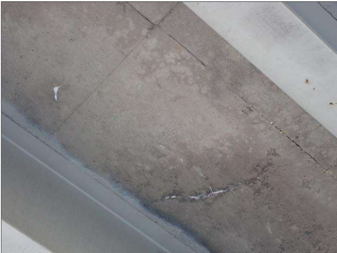
Span 3 Deck: (PAR) throughout underside of deck, in all bays, transverse cracks (up to 1/32 inch x full width) and areas of map cracks (hairline) with efflorescence buildup and rust stains
