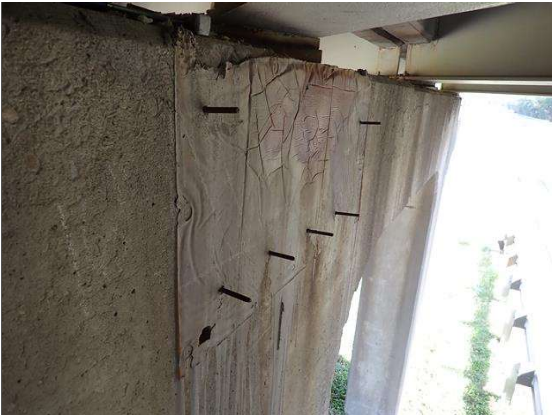
Bent 2 Cap 1: 41 inch x 23 inch patch, south face, under beam 3 with cracks up to 1/32 inch, with form bolts left in place
