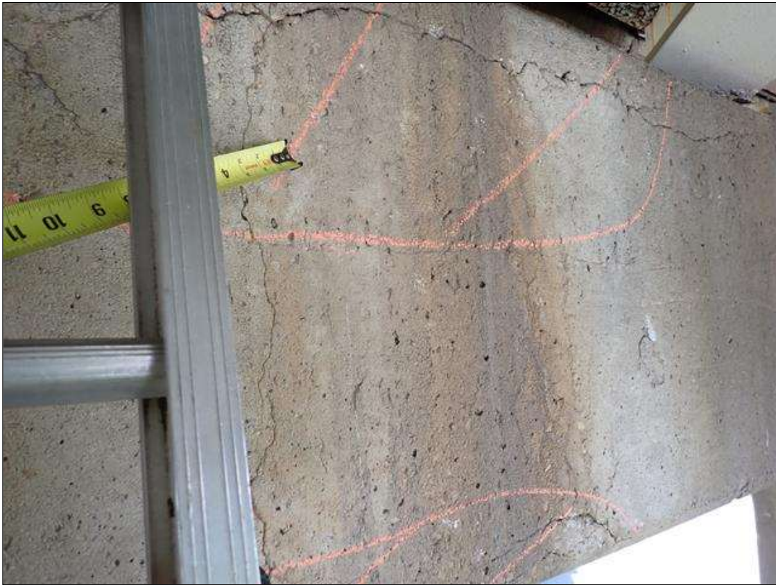
Bent 2 Cap 1: south face, below bay 3, (2) delaminations (up to 5 feet x 15 inch) with associated cracks (up to 1/16 inch)
