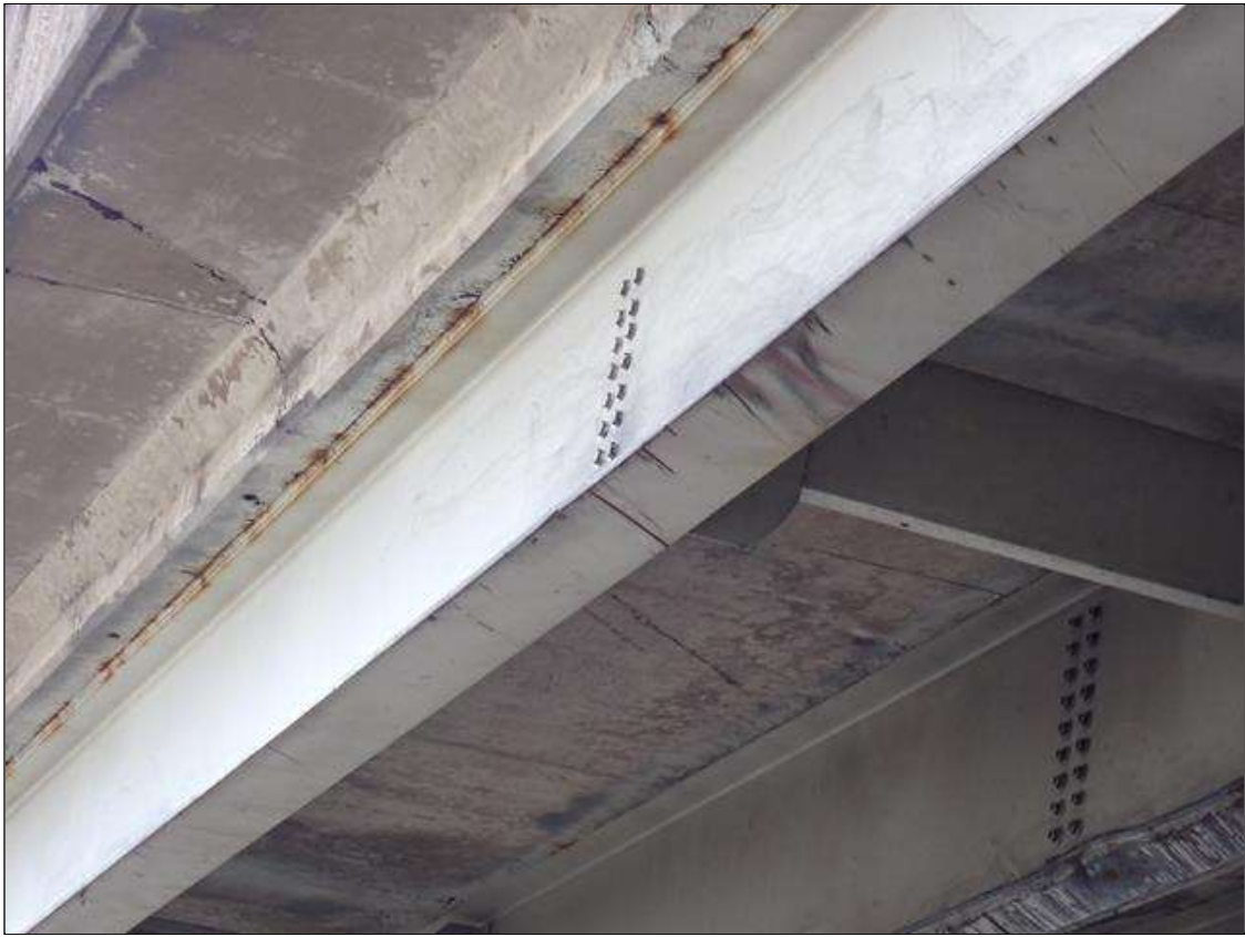
Span 2 Beam 1: impact scrapes on bottom flange with gouges up to 1/8 inch deep, 20 feet from bent 1.
