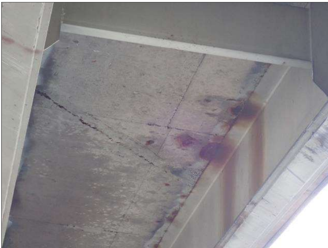
Span 3 Deck: (PAR) throughout underside of deck, in all bays, transverse cracks (up to 1/32 inch x full width) and areas of map cracks (hairline) with efflorescence buildup and rust stains
