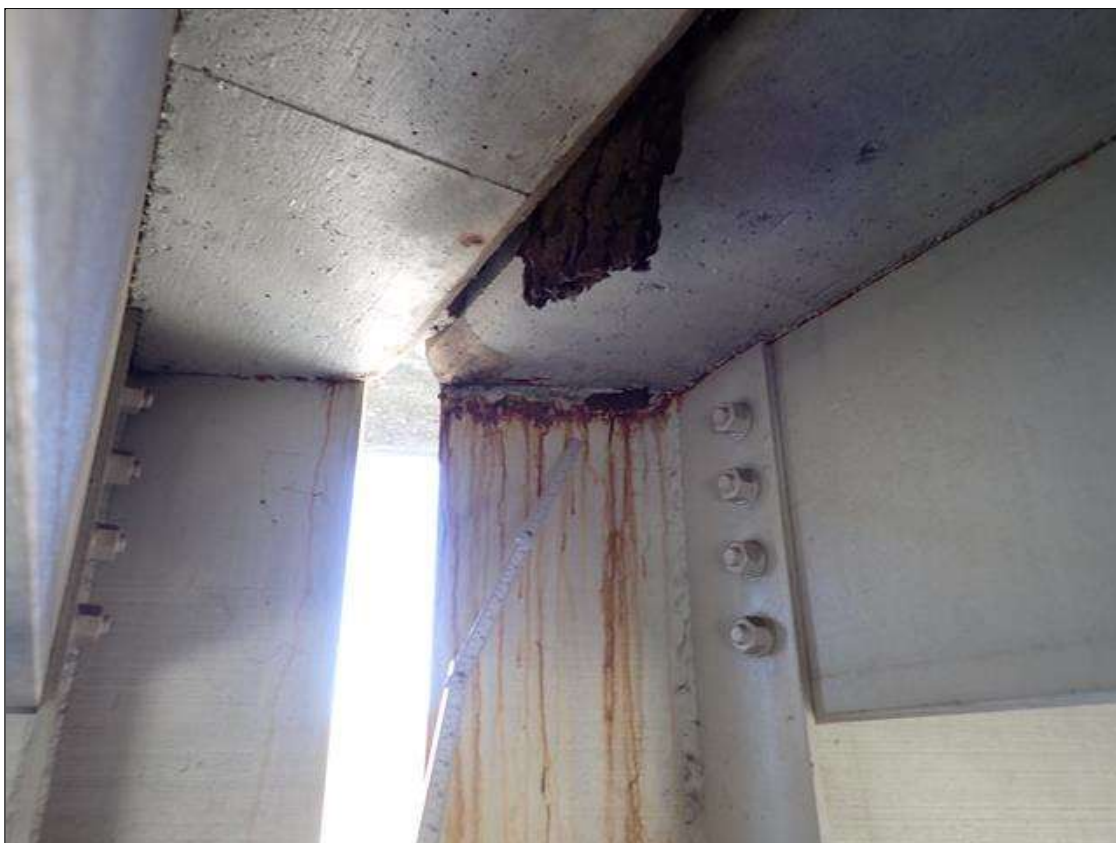
Span 3 Beam 1: at bent 2, web, rust scale (10 inch)
