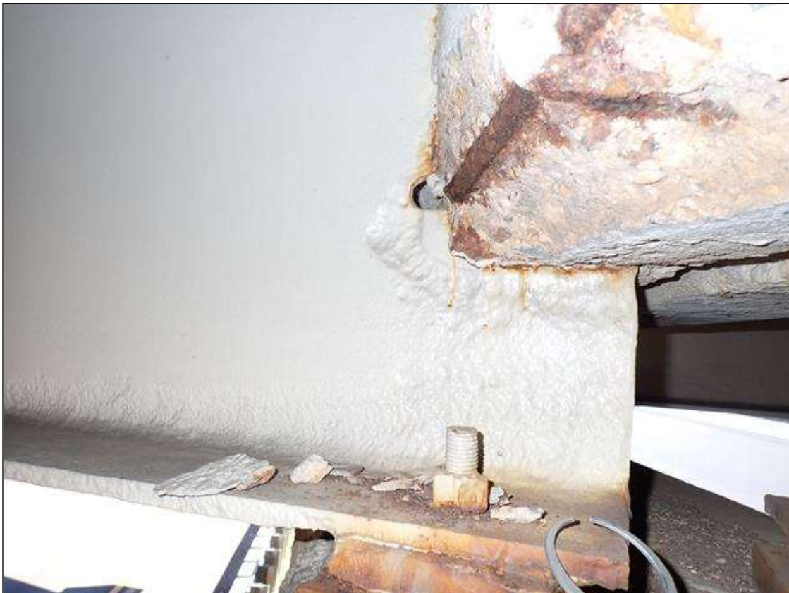
Span 3 Beam 5: (PAR) at bent 2, painted over section loss: bottom flange (0.60 inch average remaining x 3 foot); web (1/4 inch average remaining x 3 foot x 12 inch) with hole (1.5 inch x 1 inch) with corrosion reinitiated
