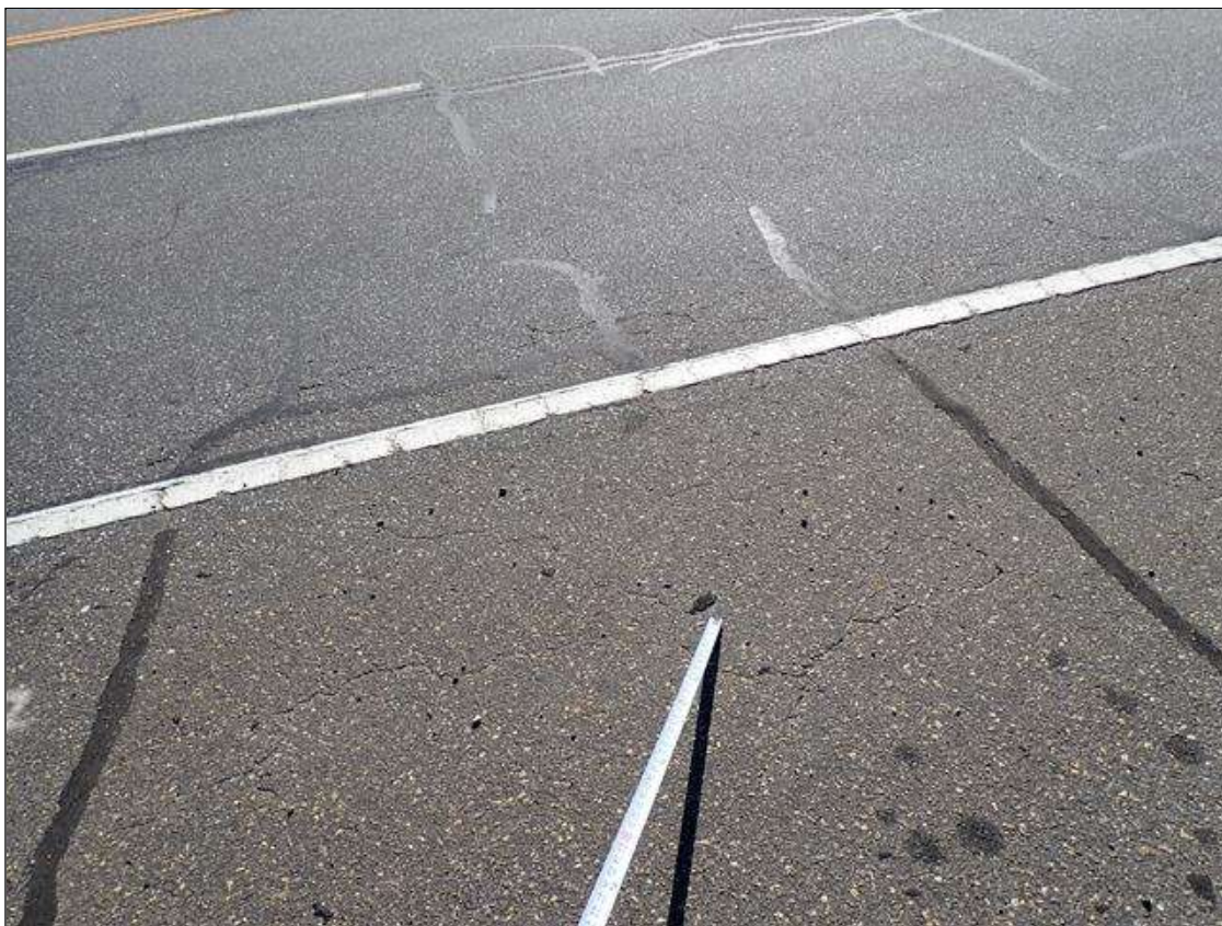
Span 2 Wearing Surface: throughout asphalt wearing surface, partially sealed transverse and longitudinal cracks (up to 1/16 inch x 8 foot)
