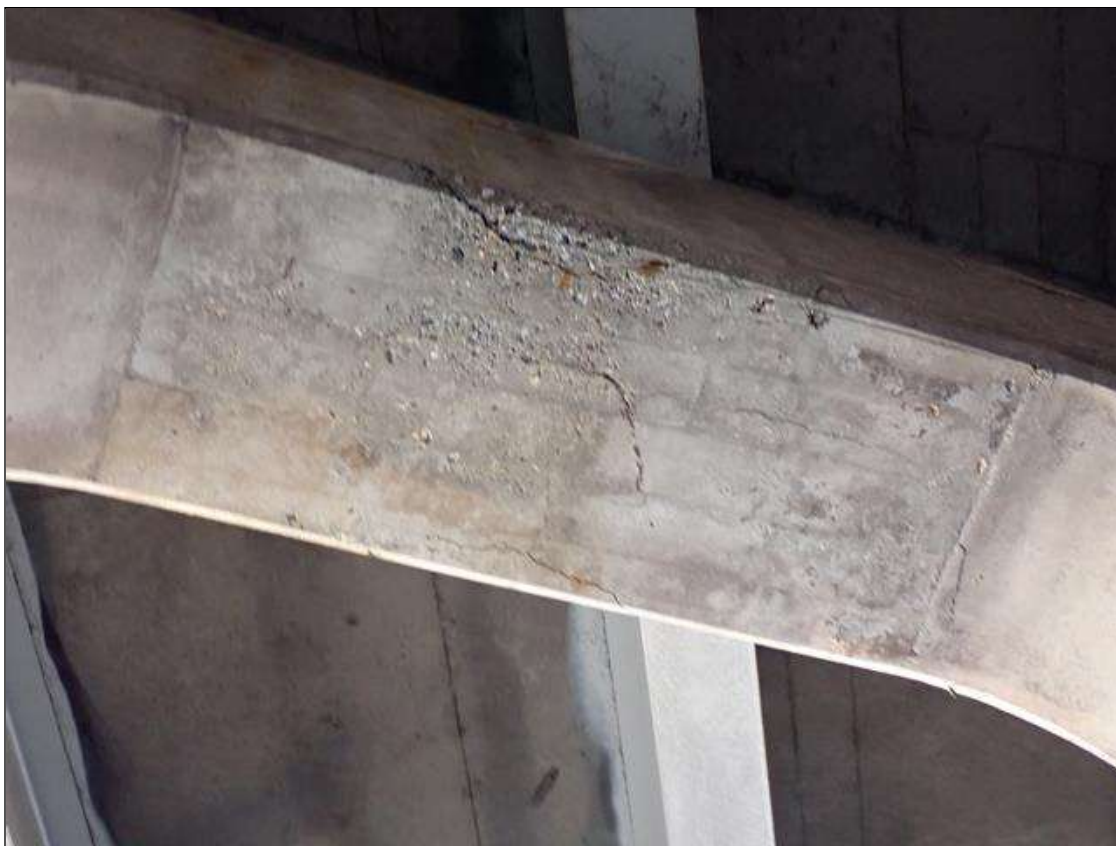
Bent 1 Cap 1: 5 foot x full width delamination with cracks up to 1/16 inch in the underside of the cap between columns 4 and 5. 1/16 inch wide vertical crack in the north face of the cap between columns 4 and 5.
