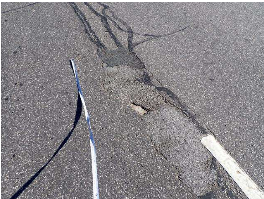
Span 1 Wearing Surface: 7 foot long x 16 foot wide x 1 inch deep failed/depresed patch in center of southbound lane near end bent 1
