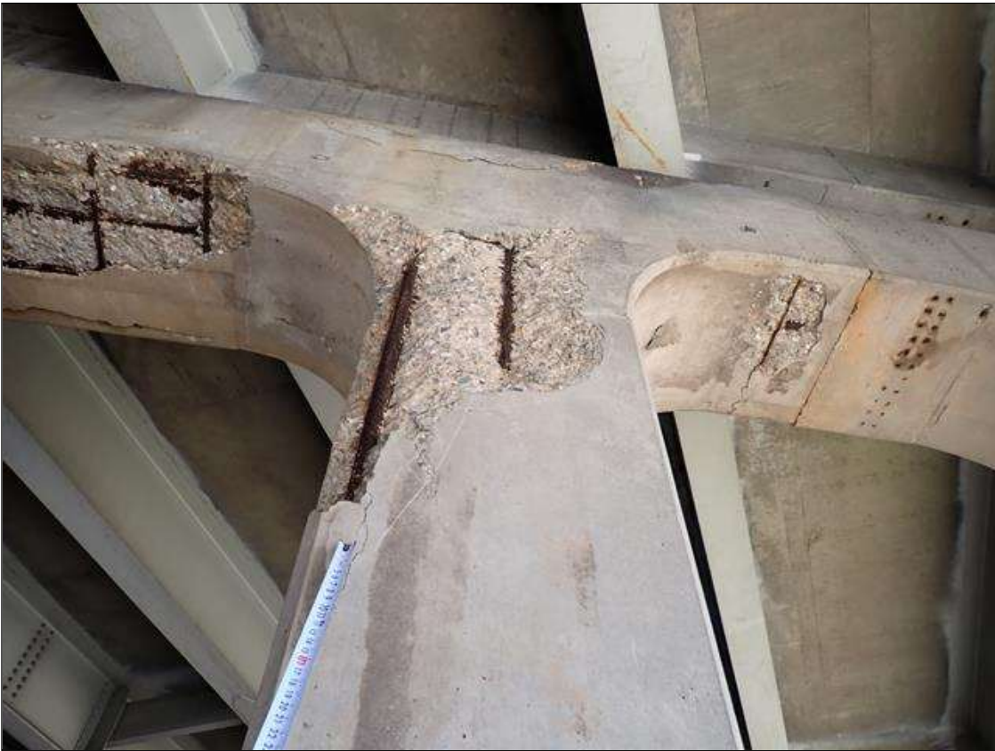
Bent 2 Pile 5: (PAR) Southwest corner below cap, delamination/spall [7 foot high x up to full width x up to 3 inch deep] with two exposed rusted reinforcing, 70 percent section remaining in the exposed reinforcement.
