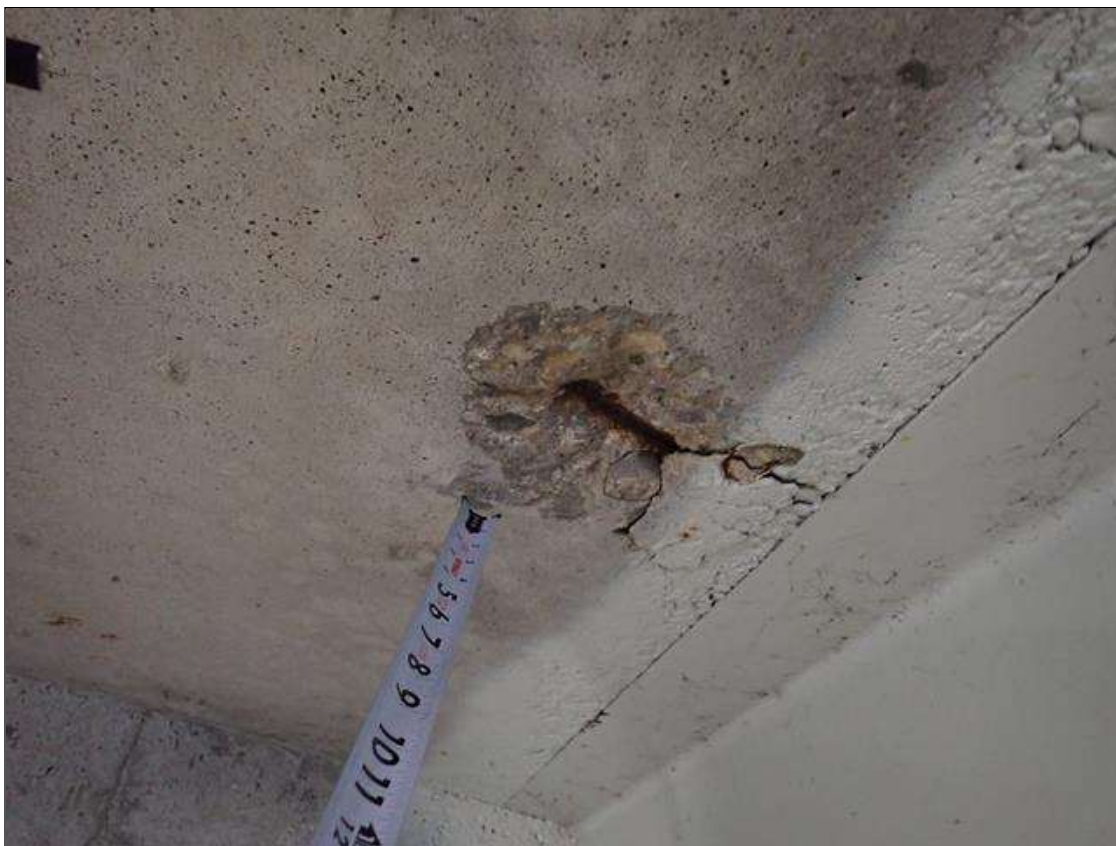
Span 1 Deck: (PAR) 6 inch diameter x 1/2 inch deep spall with exposed reinforcement in bay 4 near end bent 1
