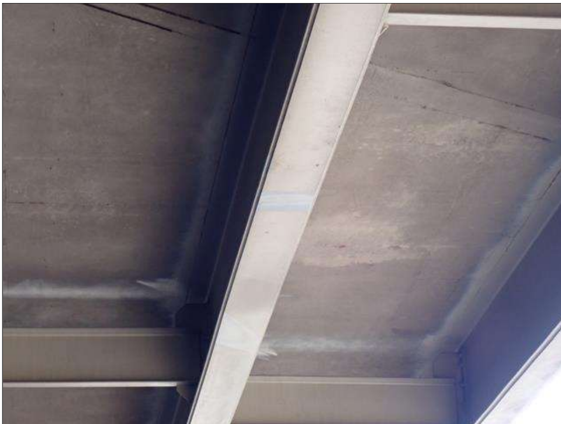
Span 3 Beam 2: 2023 new paint repair, previously noted as: SUPPLEMENTAL INSPECTION IMPACT DAMAGE 2021 :scattered scrapes
