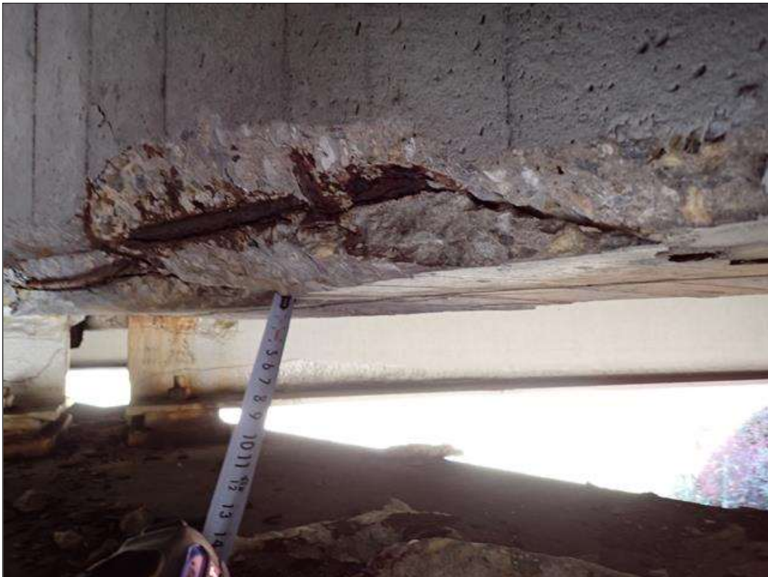
Span 2 Beam 5: (PAR) up to 4.5 foot long x 4 inch high x 3 inch deep spalls in south and bottom with exposed rusted reinforcement with up to 1/16 inch section loss, in the diaphragm between beams 4 and 5.
