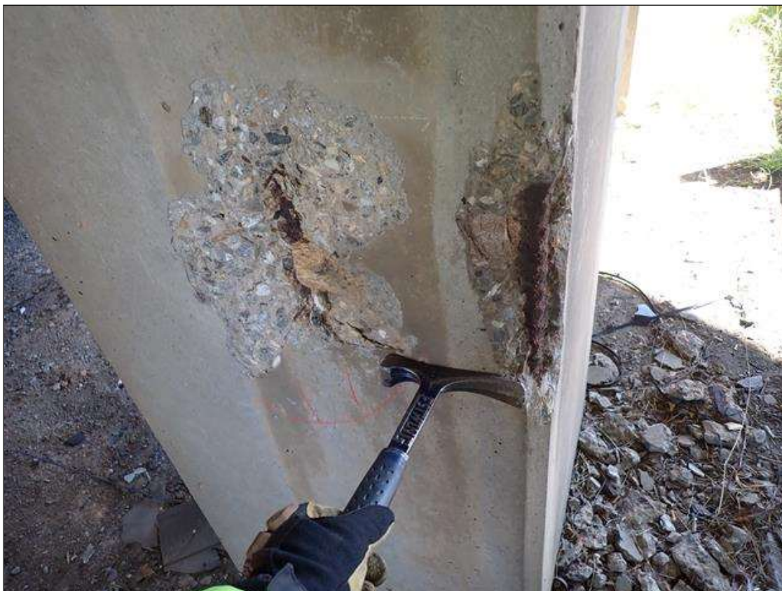
Bent 2 Pile 5: 3 foot from ground, west and south faces, (2) spalls/delaminations (up to 1 foot x 19 inch x 1.5 inch deep) with exposed rusted rebar
