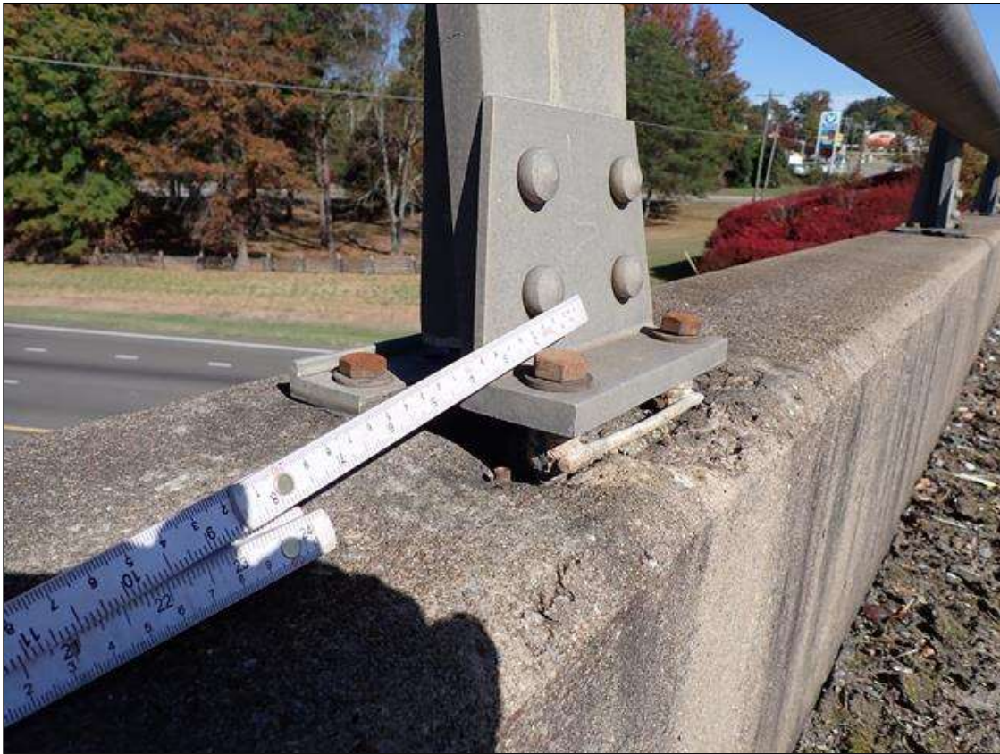
Span 2 Left Bridge Rail: (PAR) impact damage to left bridge rail at 3rd vertical post from bent 1. base plate is broken off along the weld and spalls under the base plate with two of four anchor bolts exposed. impact damage is above eastbound I-40 right travel lane. rail and post are intact
