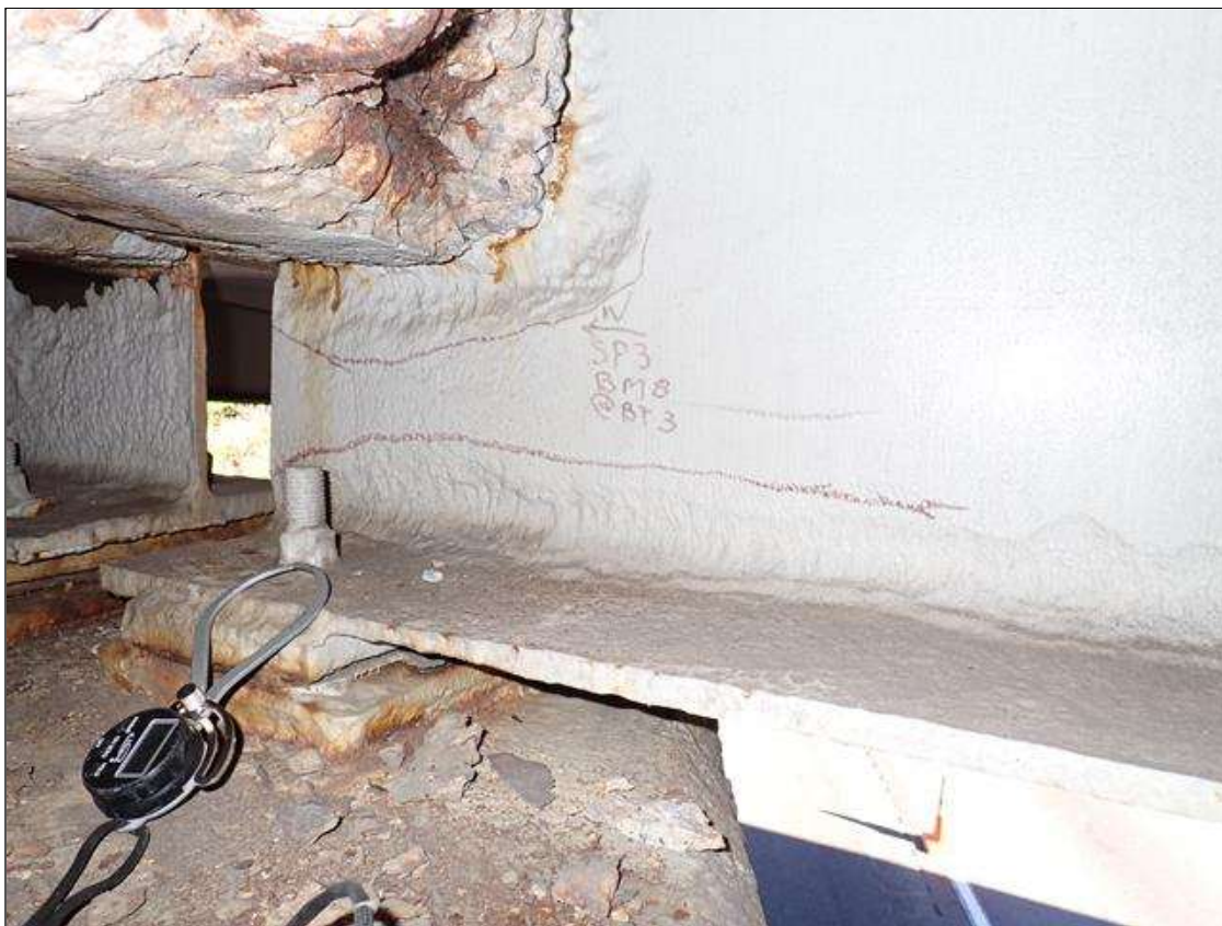
Span 3 Beam 8: (PAR) at bent 3, painted over section loss: web adjacent to diaphragm (1/4 inch average remaining x 1 foot x 8 inch); lower web (1/4 inch average remaining x 32 inch x 2 inch); bottom flange (0.50 inch average remaining x 18 inch) with corrosion reinitiated
