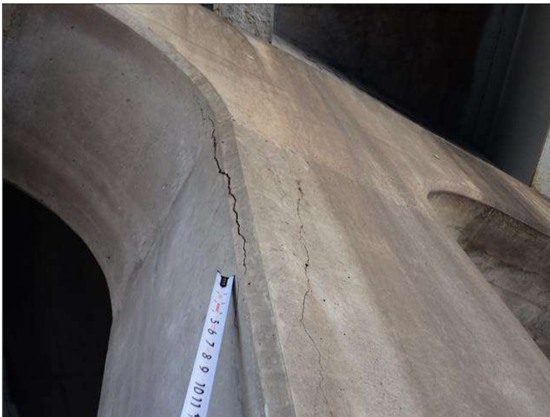
Bent 1 Pile 4: North face at top of the column, delamination [31 inch x 10 inch wide] with cracks [up to 1/8 inch]
