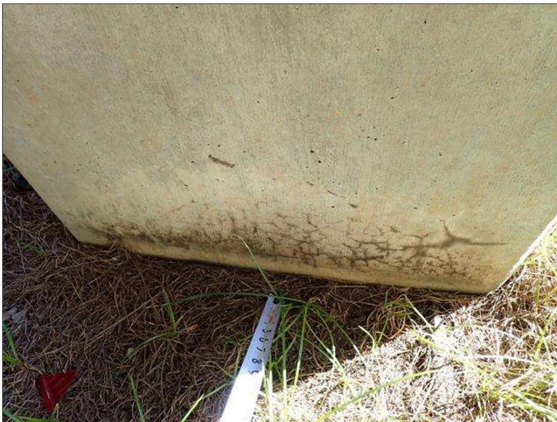
Bent 2 Pile 7: north and west faces, map cracks (hairline x 1 foot x full width)
