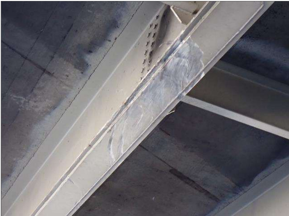
Span 3 Beam 8: over right westbound lane, impact scrapes with distortion
