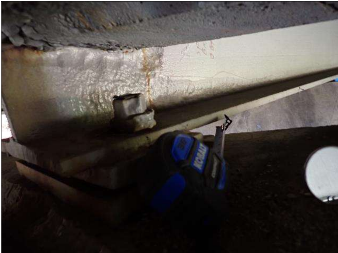
Span 4 Beam 6: (PAR) at bent 3, painted over section loss: web (1/4 inch average remaining x 32 inch x 12 inch) with corrosion reinitiated
