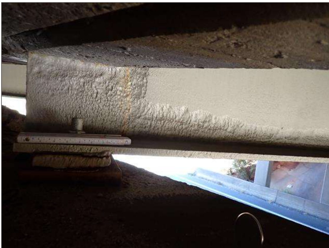
Span 3 Beam 7: (PAR) at bent 2, painted over section loss: web (1/4 inch average remaining x 4.5 foot x 16 inch)
