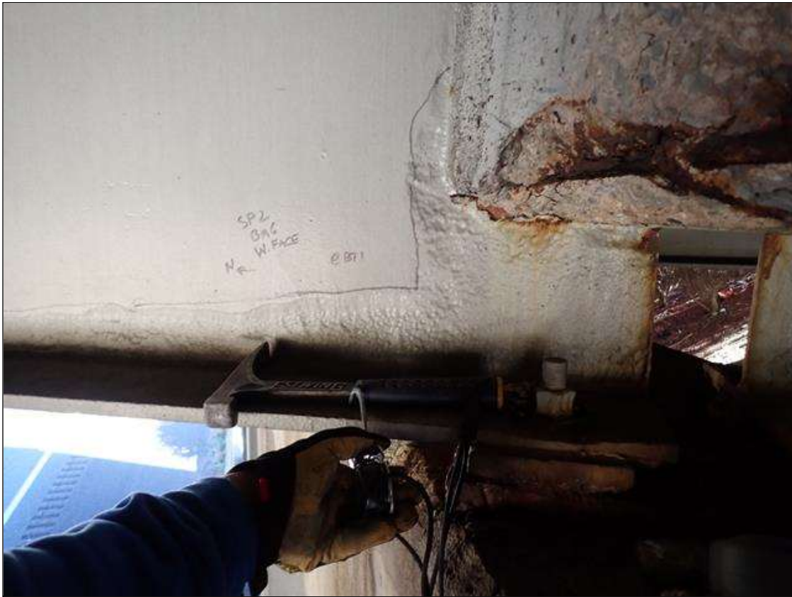
Span 2 Beam 6: (PAR) at bent 1, painted over section loss: web (1/4 inch average remaining x 54 inch x 13 inch); bottom flange (0.56 inch average remaining x 2 foot) with corrosion reinitiated
