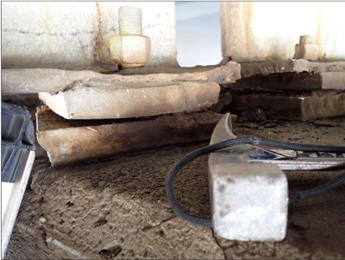
Span 2 Beam 4 - Near Bearing 4: active pack rust and section loss in masonry plate and sole plate. 75 percent section remaining
