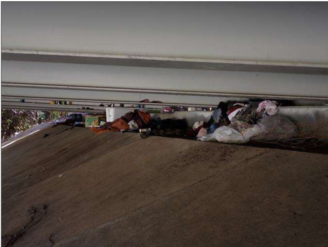
(PAR) along end bent 1 slope protection, homeless debris (full length) inhibiting inspection access
