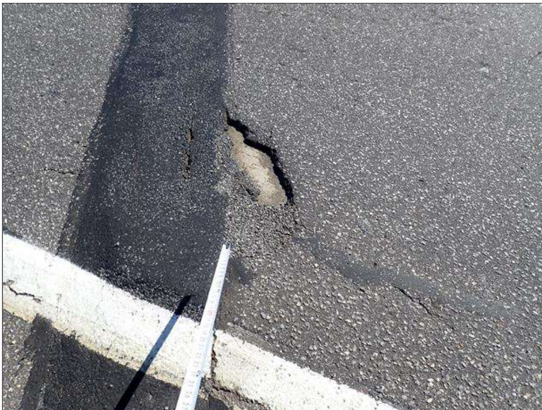
Span 2 Wearing Surface: at right Southbound lane adjacent to joint over bent 2, unsound patch/pothole [32 inch x 10 inch x full depth]
