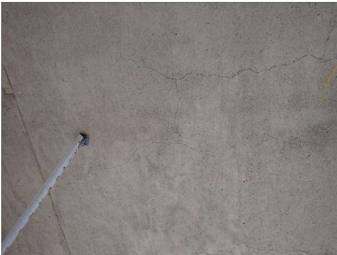
Span 1 Deck: throughout underside of deck, transverse cracks (up to 1/16 inch x full bay width) and map cracks (1/32 inch) at random
