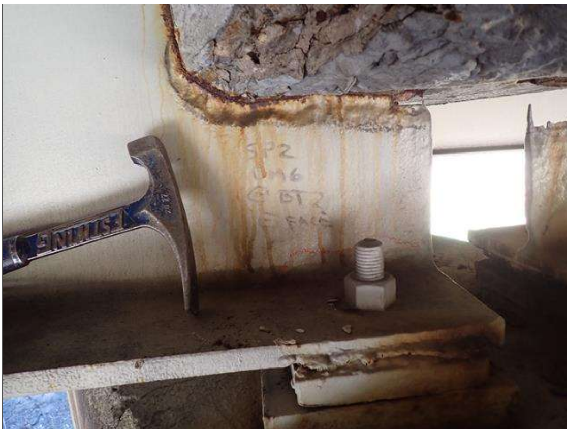
Span 2 Beam 6: (PAR) at bent 2, painted over section loss: web adjacent to diaphragm (3/16 inch average remaining x 10.5 inch x 2.5 inch) with corrosion hole (1.5 inch x 1/2 inch); lower web (3/8 inch average remaining x 5.5 inch x 1 inch) with corrosion reinitiated
