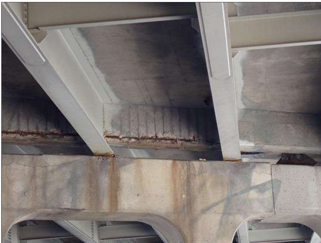
Span 3 Beam 4: (PAR) 6 foot long x up to 3 inch high x 10 inch wide area of spall in the diaphragm between beams 4 and 5 at bent 2 with exposed reinforcement. 70 percent section remaining in the exposed reinforcement.
