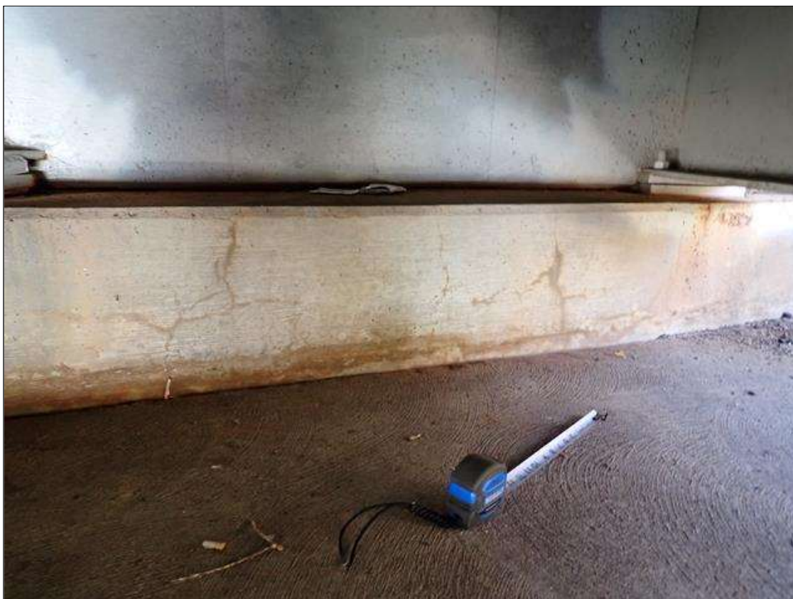
End Bent 1 Cap 1: west end, map cracks (hairline x 1.5 foot x full height)
