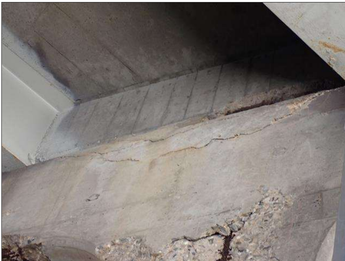
Bent 2 Cap 1: 4 foot long x 18 inch x 1 inch high spall/delamination concrete in south face near the top between beams 7 and 8.
