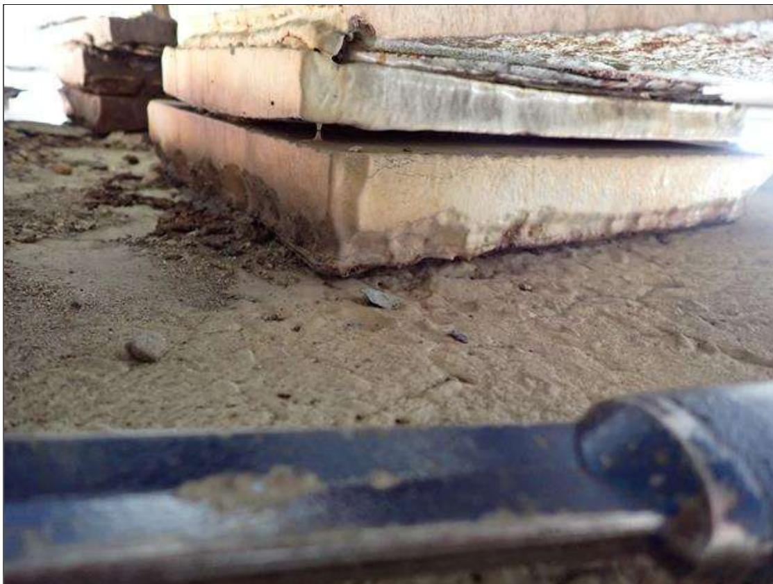
Span 2 Beam 5 - Far Bearing 5: painted over section loss (up to 1/8 inch loss) on masonry plate and sole plate
