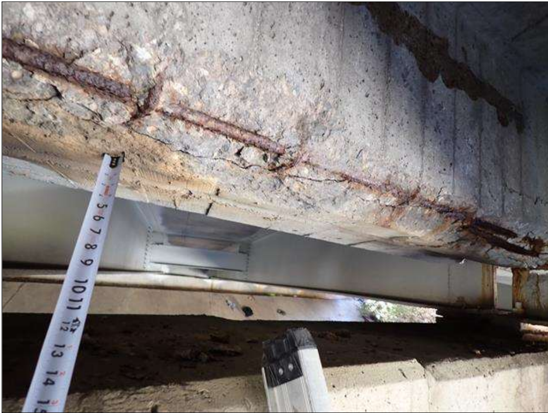
Span 2 Beam 4: (PAR) 7 foot long x 4 inch high x 4 inch wide area of spall, delamination with exposed reinforcement in the concrete diaphragm between beams 4 and 5 at bent 1. 75 percent section remaining in the exposed reinforcement.
