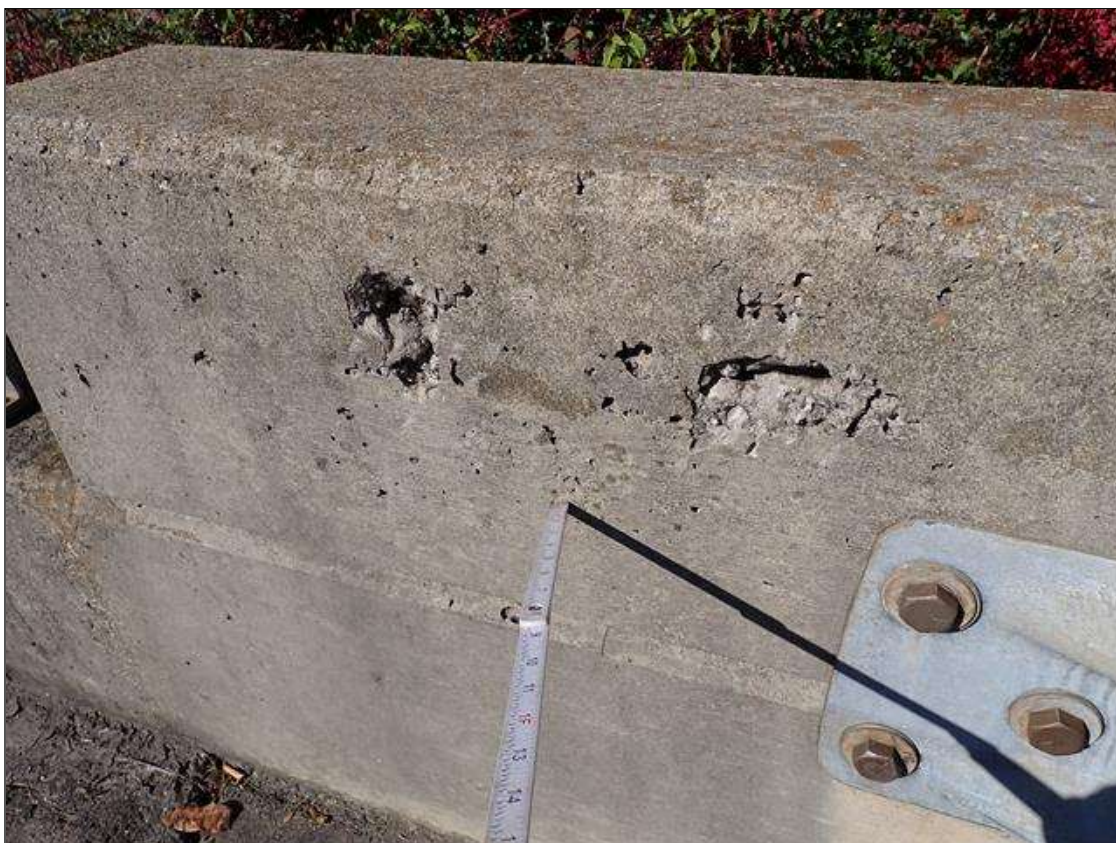
Span 4 Left Bridge Rail: at end bent 2, (2) spalls (up to 5 inch x 4 inch x 1.5 inch deep) exposed reinforcement. no measureable section loss.
