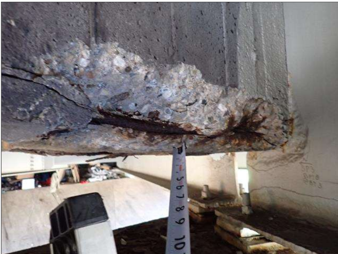
Span 3 Beam 8: (PAR) 3 foot long x 6 inch wide x 3 inch high spall with exposed reinforcement in end diaphragm between beams 7 and 8 at bent 3. 70 percent section remaining in exposed reinforcement.
