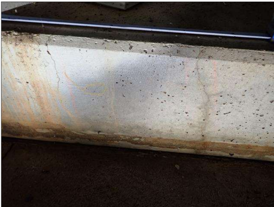
End Bent 1 Cap 1: scattered along length of cap, multiple vertical cracks [15 inch long x up to 1/32 inch]
