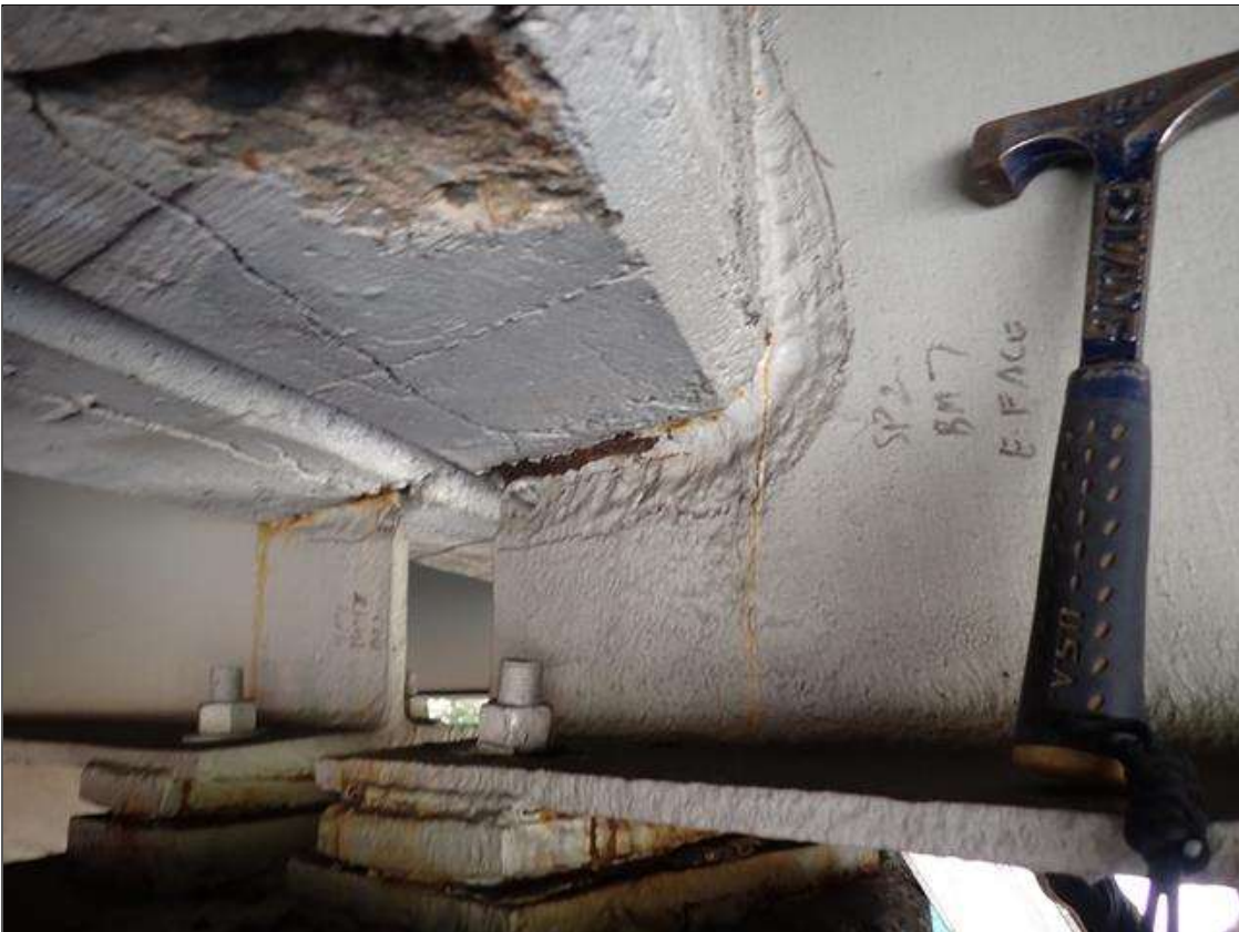
Span 2 Beam 7: (PAR) at bent 1 active corrosion with section loss, web at diaphragm [20 inch long x 13 inch high x 1/4 inch average remaining] with multiple corrosion holes up to [3 inch x 1 inch]
