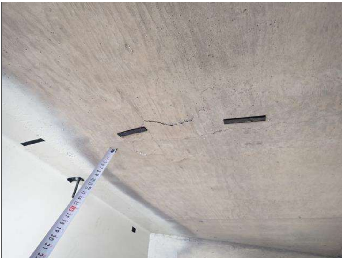
Span 1 Deck: underside of deck, bay 2, at end bent 1 and midspan, (2) delaminations (up to 3 foot x 1 foot)
