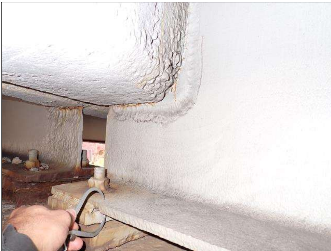
Span 2 Beam 5: (PAR) at bent 2, painted over section loss: bottom flange (0.50 inch average remaining x 8 inch); web adjacent to diaphragm (3/16 inch average remaining x 11 inch x 8 inch) with corrosion reinitiated
