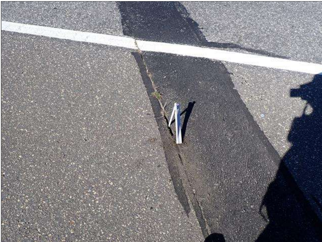
Span 4 Expansion Joint at Bent 3: along the length of the joint, adhesion loss (up to 3/4 inch wide x 7 foot x 1.5 inch deep) at random
