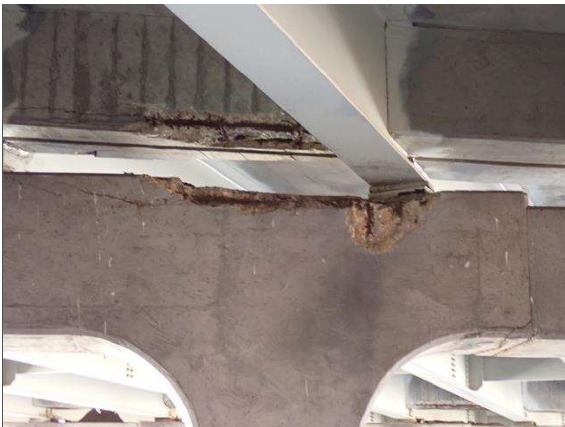
Bent 1 Cap 1: (PAR) South and top face between beams 7 and 8, spall/delamination [4.5 foot x up to 3.5 foot x up to 4 inch deep] with 4 vertical and 1 horizontal exposed rusted reinforcing with up to 1/16 inch section loss. no loss of bearing area
