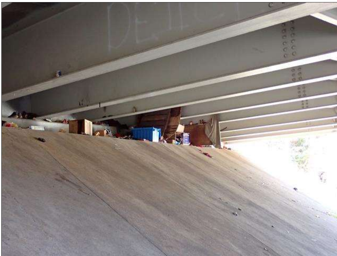
(PAR) along end bent 2 slope protection, homeless debris with inhabitants (full length) inhibiting inspection access
