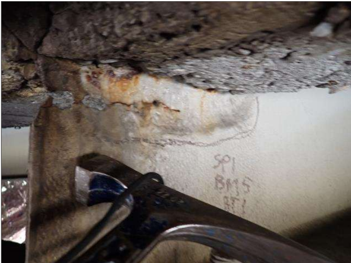
Span 1 Beam 5: (PAR) 10 inch long x 3 inch high x 3/16 inch average remaining in the web with 3 inch long x 1.5 inch corrosion hole under the diaphragm at bent 1
