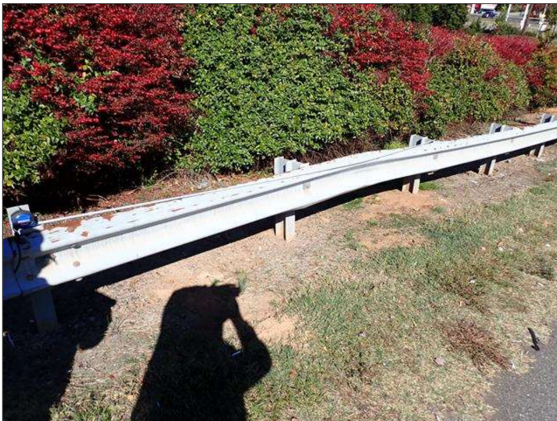
(PAR) northwest guardrail, 55 foot from end bent 2, impact damage (12.5 foot)
