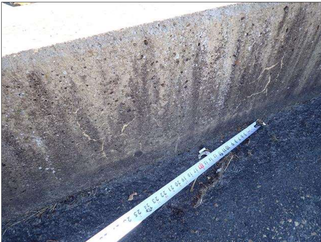
Span 3 Right Bridge Rail: adjacent to rail post 6, hairline map cracking
