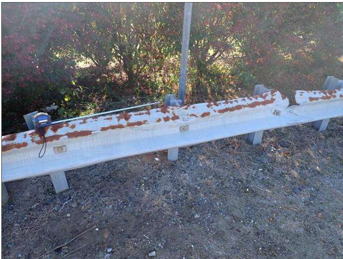
(PAR) southeast guardrail, 3 foot from end bent 1, impact damage (9 foot)
