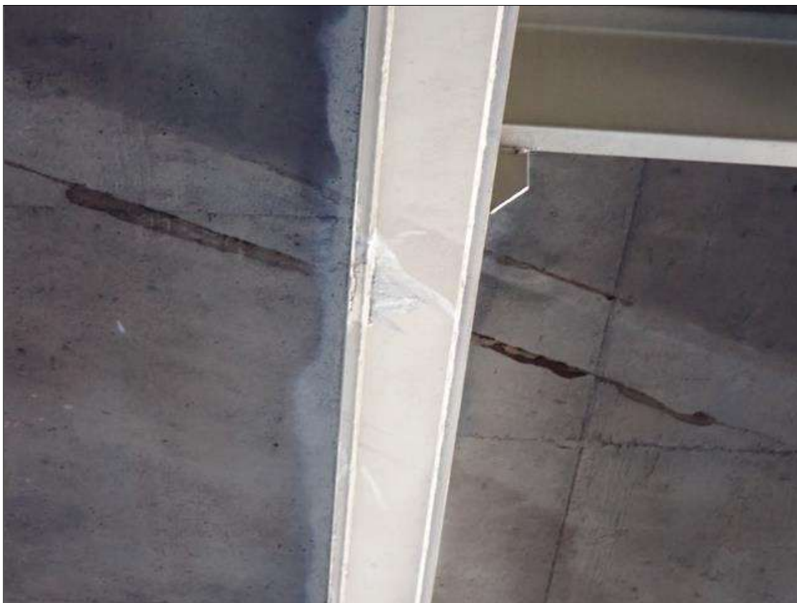
Span 3 Beam 7: over right westbound lane, impact scrapes
