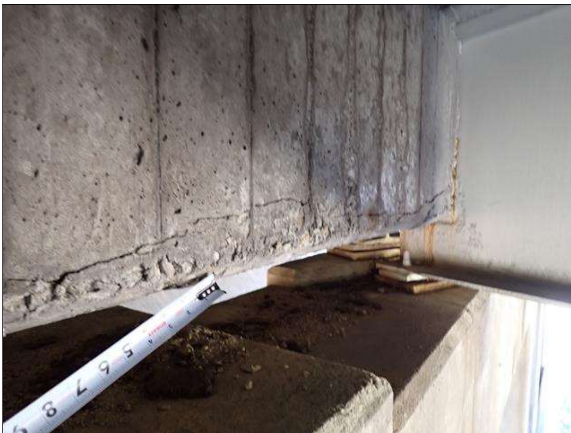
Span 3 Beam 5: 7 foot x 4 inch delamination with cracks up to 1/8 inch in south face end diaphragm at bent 3
