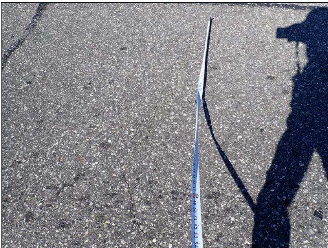
Span 1 Wearing Surface: throughout asphalt wearing surface, partially sealed transverse and longitudinal cracks (up to 1/16 inch x 8 foot)
