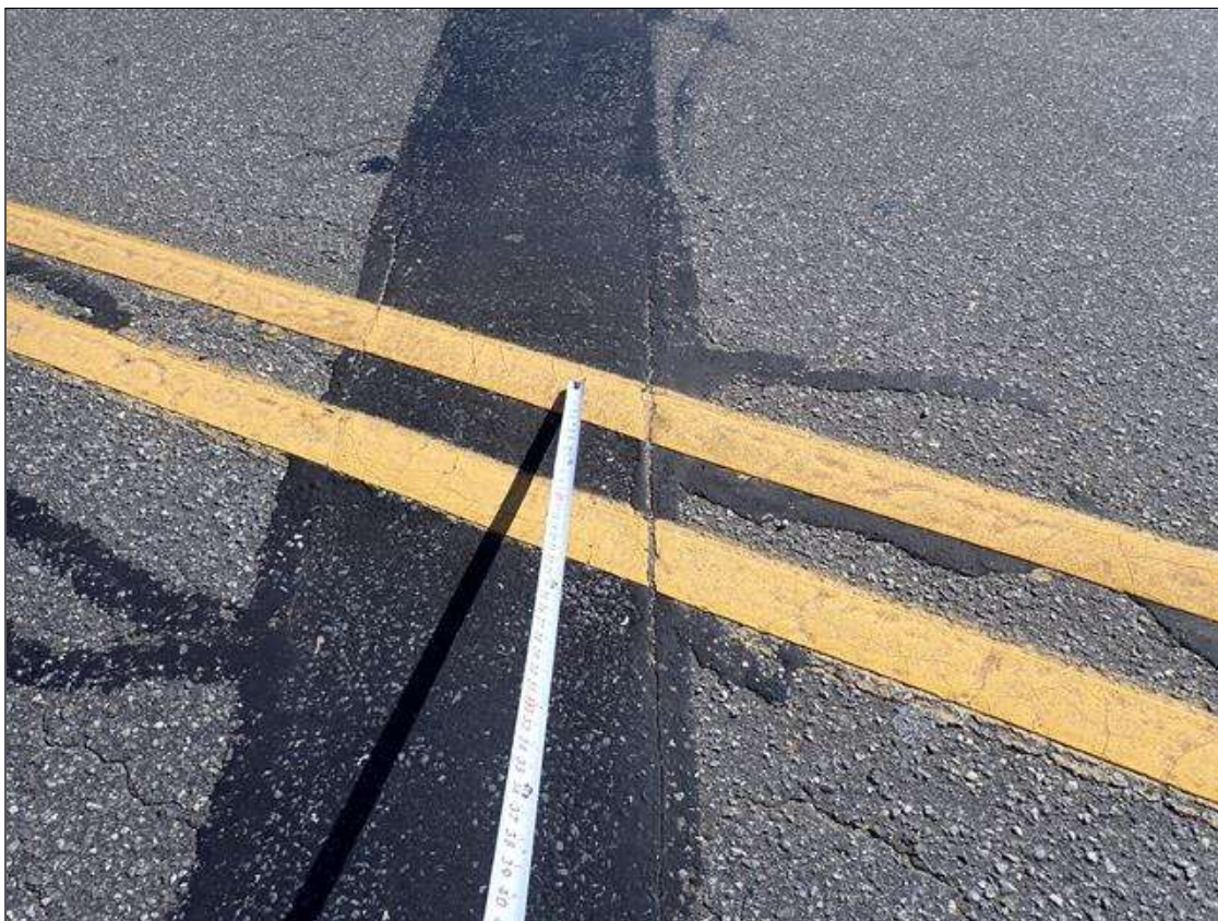
Span 3 Expansion Joint at Bent 2: along the length of the joint, adhesion loss (up to 1/8 inch wide x 2.5 foot x 3/4 inch deep) at random
