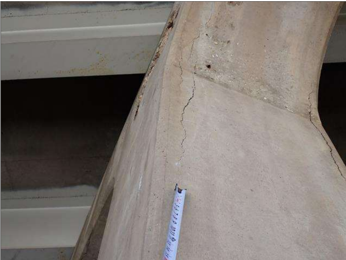
Bent 2 Pile 4: below cap, northeast and southeast corners, (2) delaminations (up to 3.5 foot x 10 inch) with cracks (1/4 inch)
