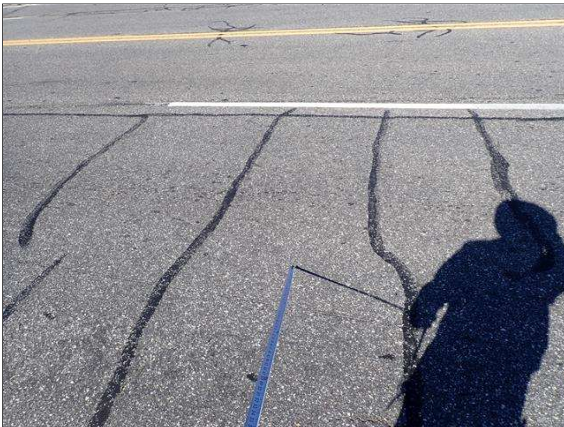
Span 1 Wearing Surface: throughout asphalt wearing surface, partially sealed transverse and longitudinal cracks (up to 1/16 inch x 8 foot)
