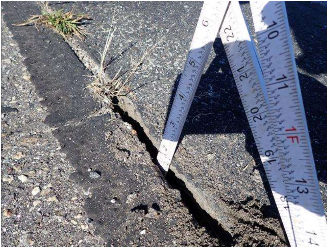
Span 4 Expansion Joint at Bent 3: along the length of the joint, adhesion loss (up to 3/4 inch wide x 7 foot x 1.5 inch deep) at random
