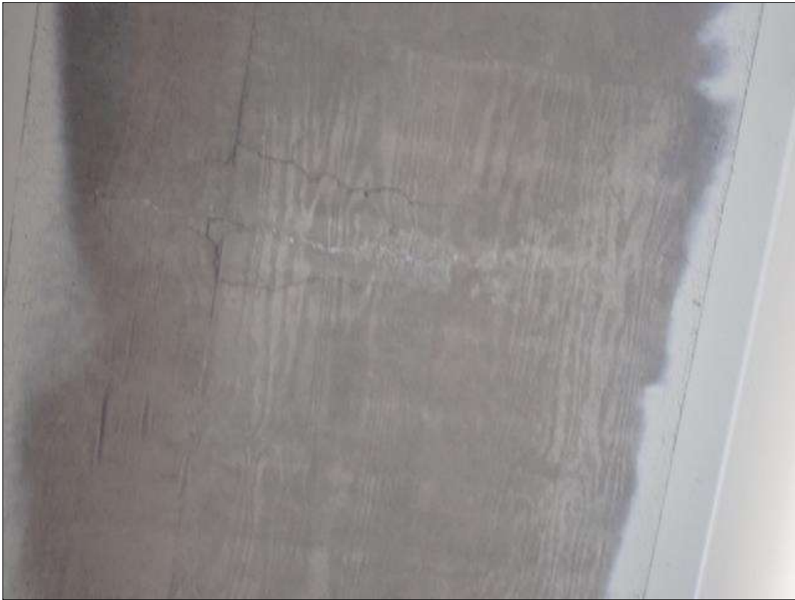
Span 1 Deck: (2) up to 2 foot wide x 12 inch long areas of delamination in deck underside, bay 3, near midspan.
