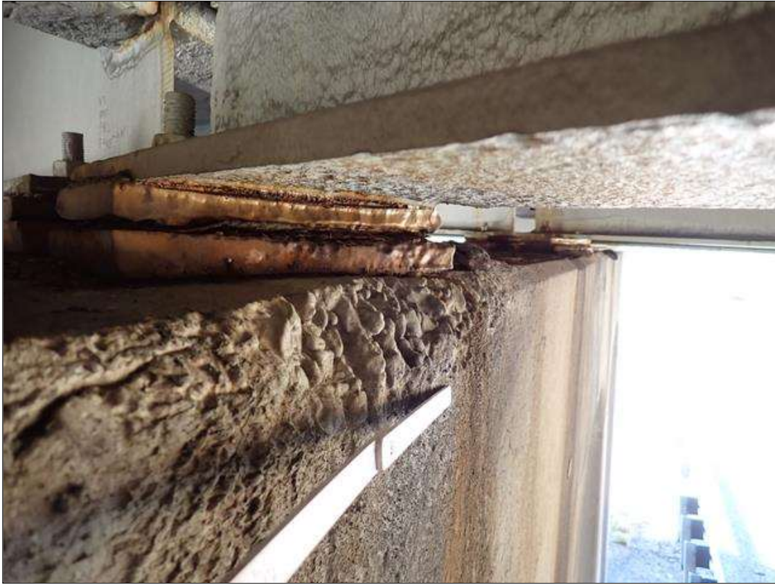
Bent 2 Cap 1: under beam 5, spall [14 inch x 4 inch x 1 inch deep] with coarse aggregate exposed, undermining bearing 1/2 inch
