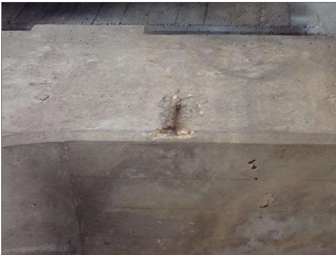
Bent 3 Cap 1: 10 inch x 5 inch x 1 inch deep spall with exposed reinforcement in south face between beams 6 and 7. 90 percent section remaining in exposed reinforcement.
