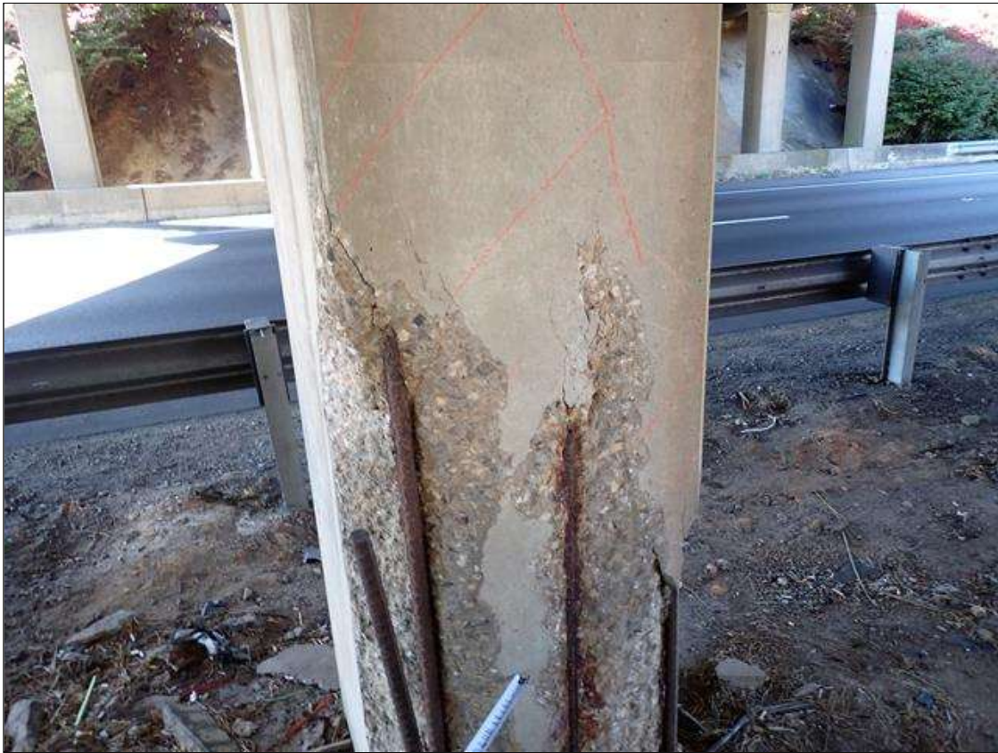
Bent 2 Pile 4: (PAR) north face, at ground, spall/delamination (full width x 7.5 foot high x 3 inch deep) extends into east and west faces (up to 7 inch) with exposed rusted and debonded rebars
