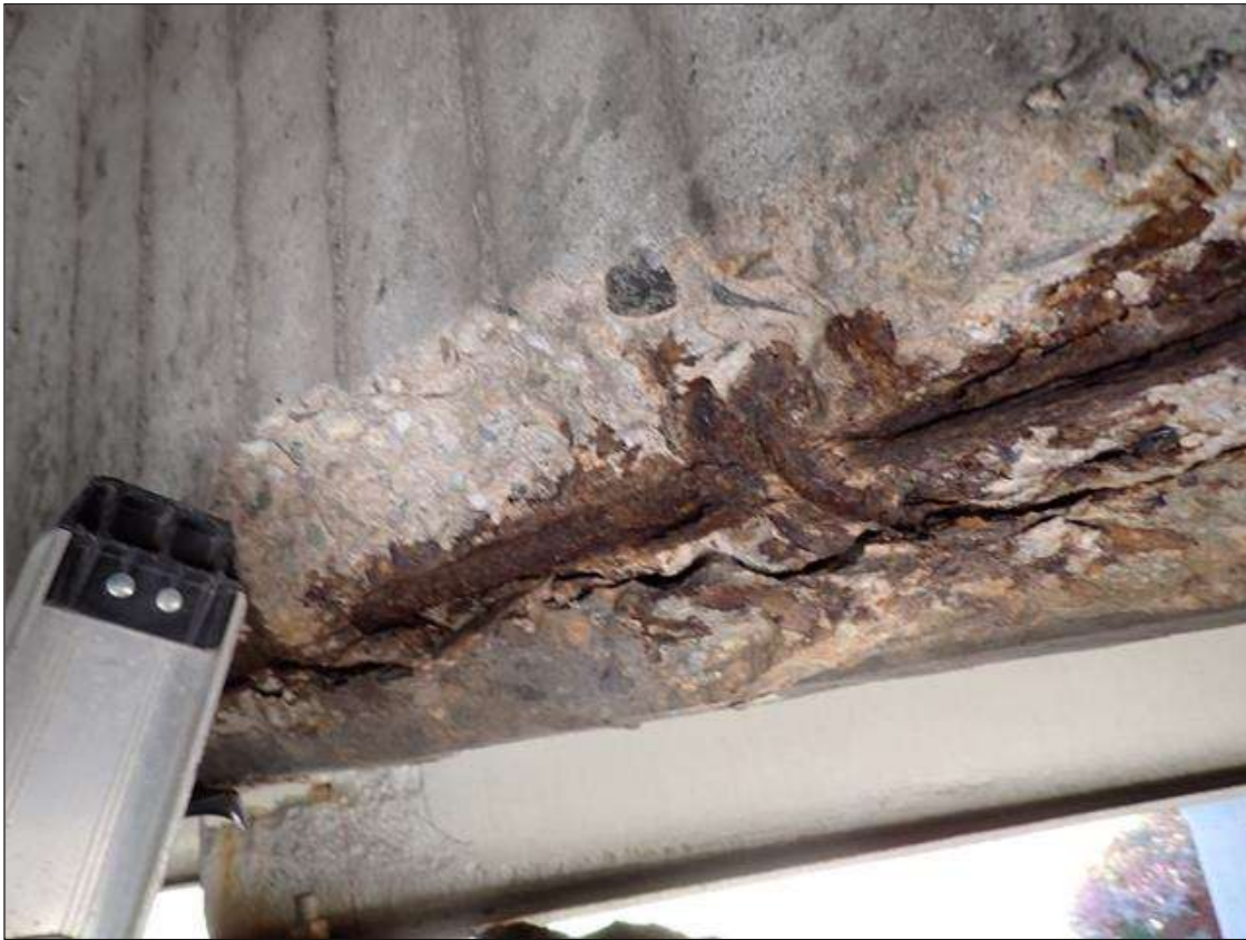
Span 2 Beam 6: (PAR) 7 foot x 16 inch x up to 3 inch deep spall with exposed reinforcement in the underside and south face of the diaphragm between beams 6 and 7. 70 percent section remaining in exposed reinforcement.
