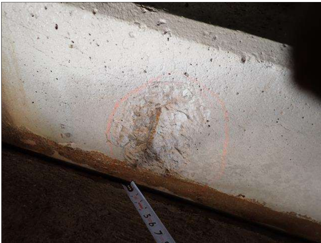
End Bent 1 Cap 1: 11 inch high x 7 inch wide x up to 1 inch deep spall with exposed rusted rebar in north face of cap at beam 4.
