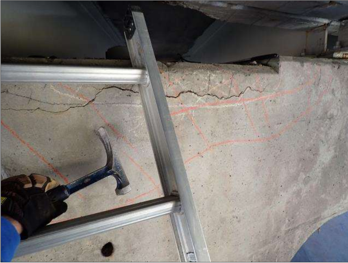
Bent 1 Cap 1: 5 foot long x 21 inch high area of delaminated concrete with cracks up to 1/16 inch between beams 7 and 8 in the north face of cap near top.
