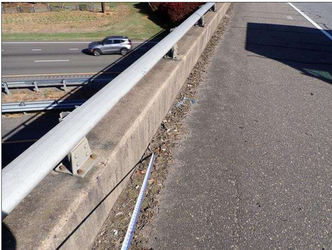
along both curblines, debris accumulation (1 foot wide x full length); partially obstructing deck drainage
