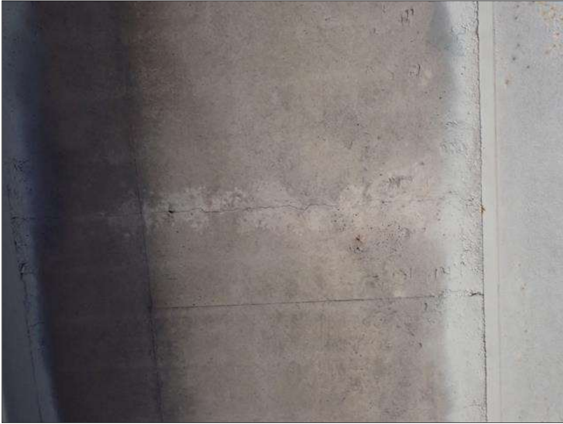
Span 2 Deck: throughout underside of deck, transverse cracks (up to 1/16 inch x full bay width) and map cracks (1/32 inch) at random
