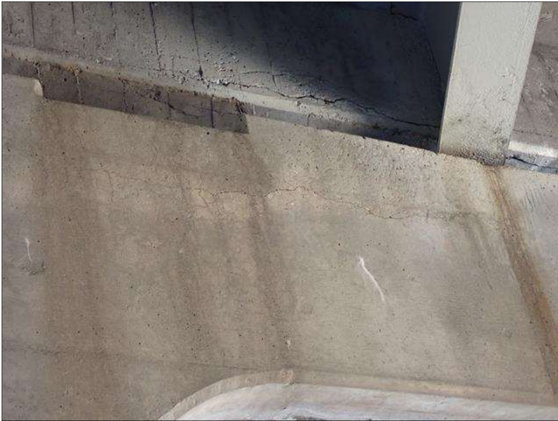
Bent 3 Cap 1: 4 foot long x 8 inch high area of up to 1/16 inch wide cracks and delamination on north face under bay 5
