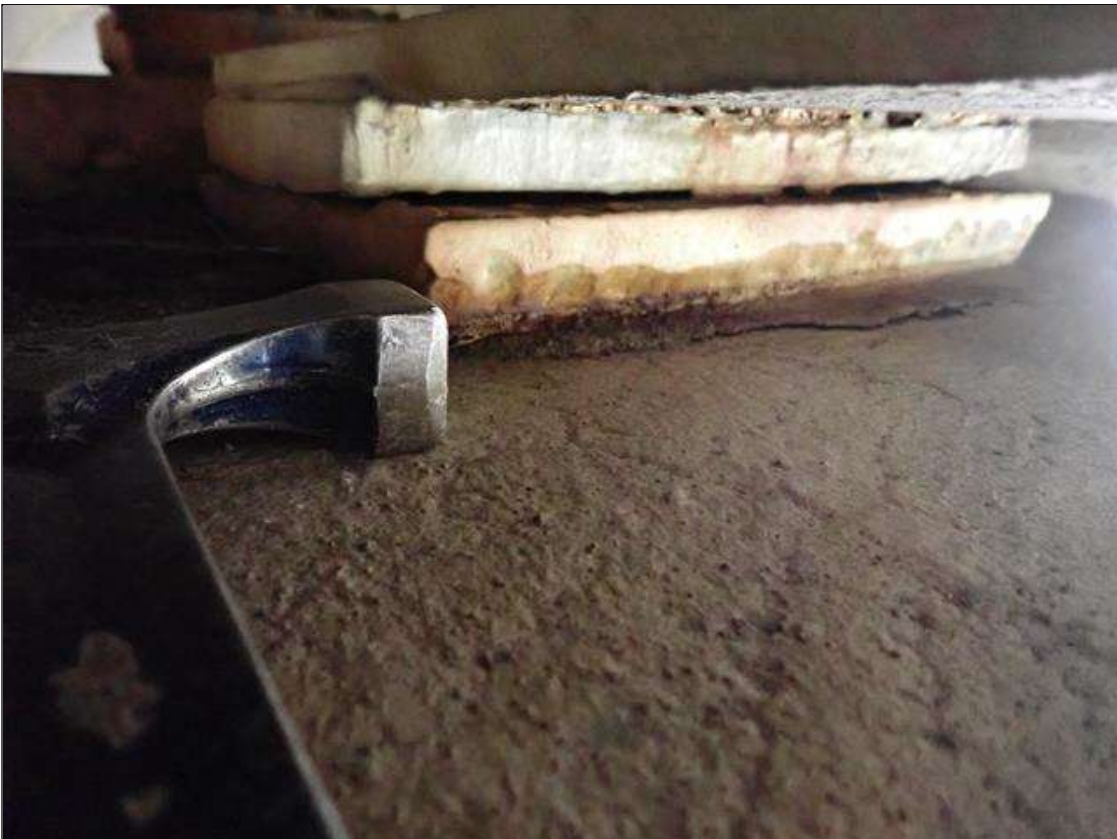
Span 3 Far Bearing 7: arrested pack rust and section loss in masonry plate and sole plate. 80 percent section remaining.
