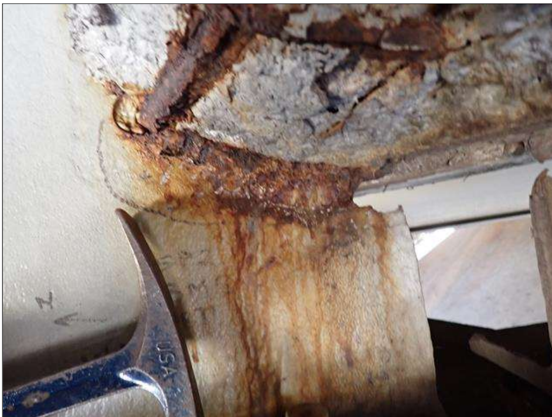
Span 2 Beam 5: (PAR) active corrosion with section loss 10 inch long x 3 inch high x 1/4 inch average remaining in the web with 3 inch long x 1.25 inch high corrosion hole under the diaphragm at bent 1
