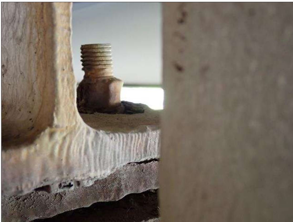
Span 4 Beam 7 - Near Bearing 7: arrested corrosion and section loss in masonry plate and sole plate. 80 percent section remaining. both anchor bolt nuts have up to 40 percent section remaining
