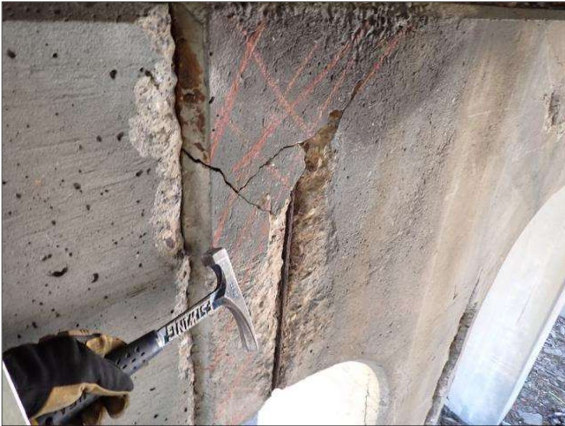
Bent 2 Cap 1: (PAR) south face, below beam 4, spall/delamination (18 inch x 38 inch x 1.5 inch deep) with exposed and debonded rebar
