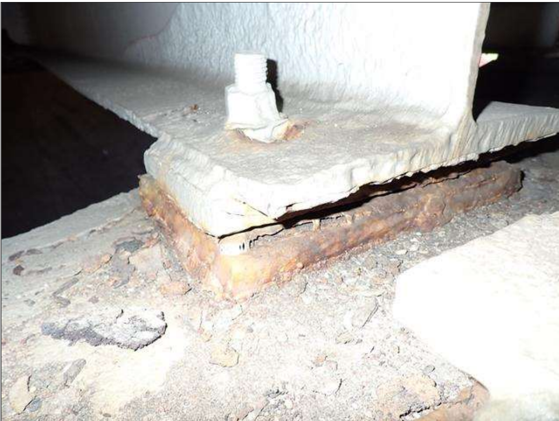
Span 4 Beam 8 - Near Bearing 8: corrosion has been arrested when painted, 75 percent section remaining in masonry plate and sole plate. both anchor bolt nuts have up to 50 percent section remaining.
