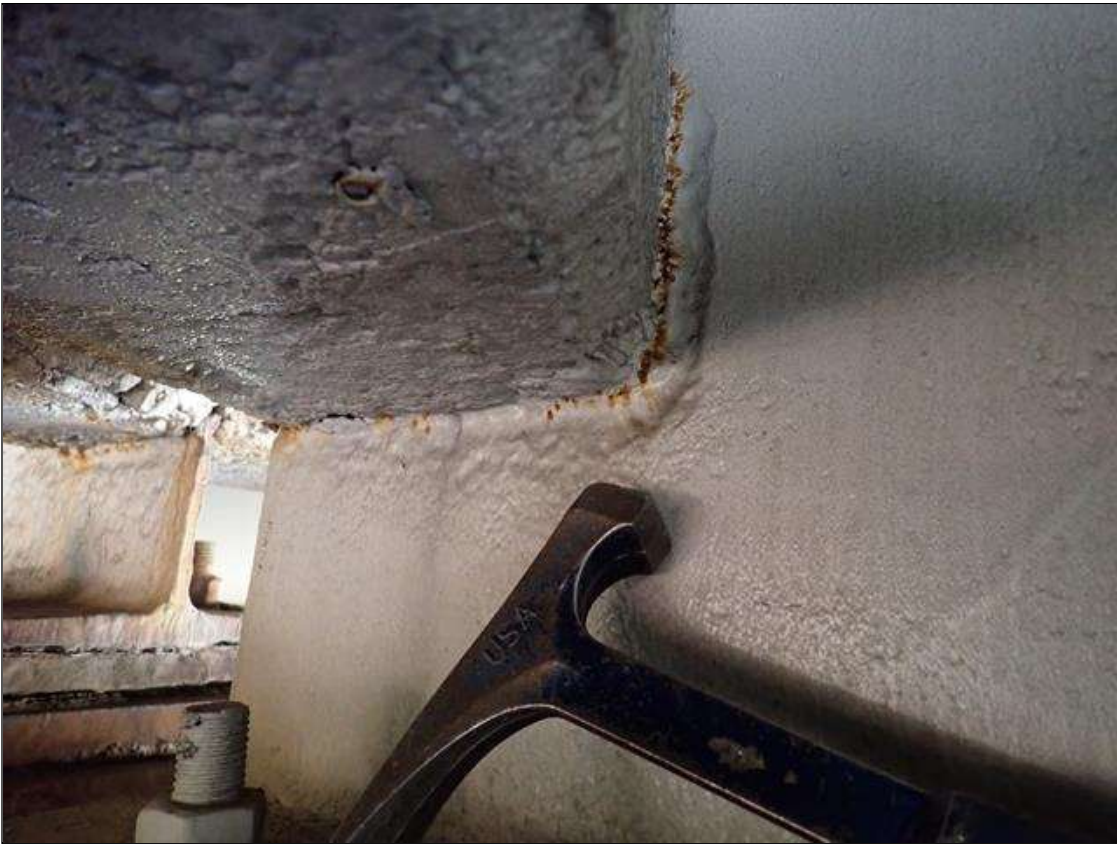
Span 3 Beam 7: (PAR) at bent 3, painted over section loss: web adjacent to diaphragm (3/8 inch average remaining x 10 inch x 5 inch) with corrosion reinitiated
