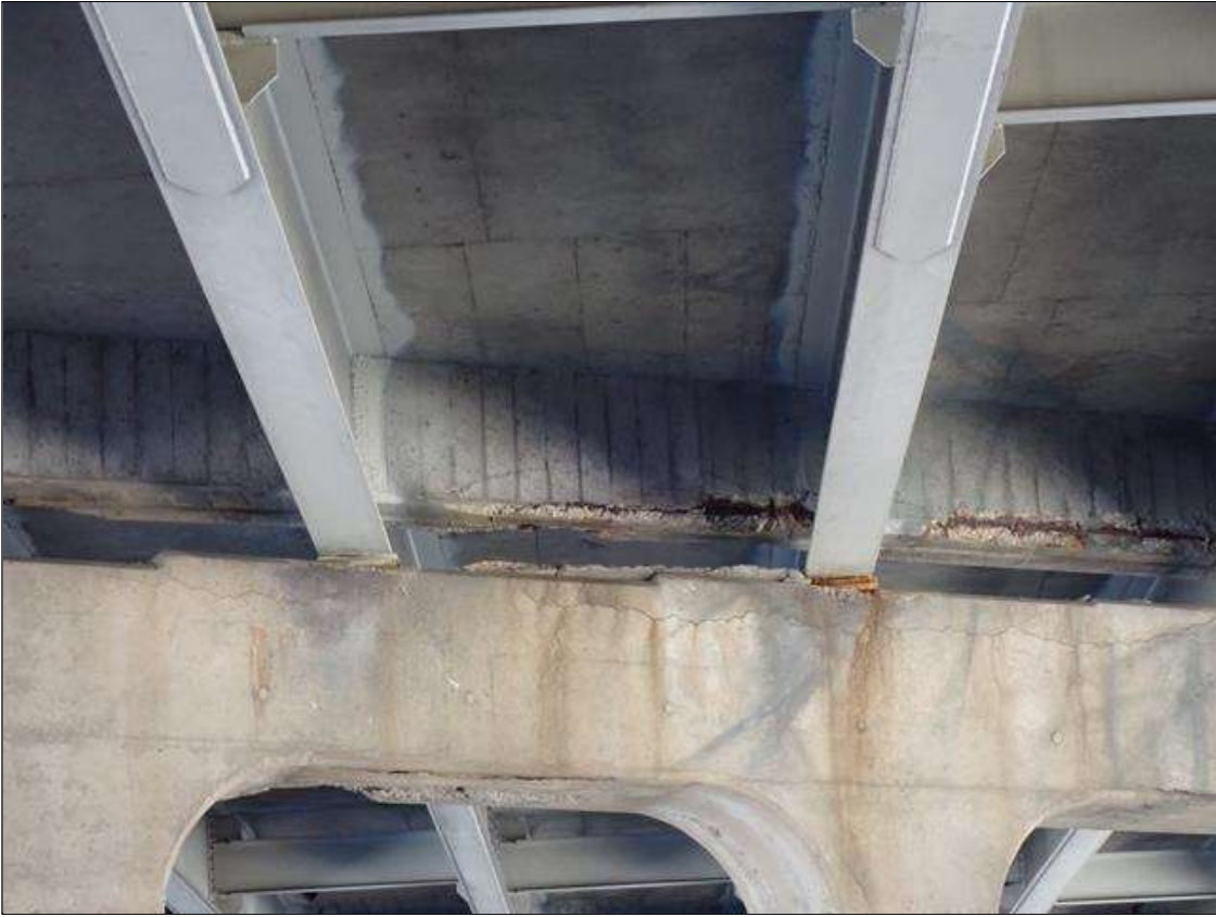
Span 3 Beam 6: spall/delamination 7 foot x 10 inch x 2 inch deep with exposed rusted rebar in north face of end diaphragm between beams 6 and 7 at bent 2
