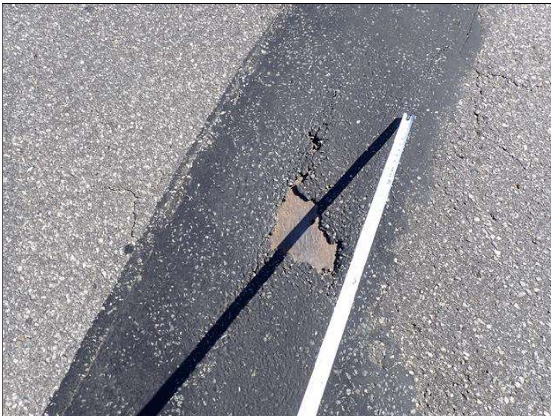
Span 2 Expansion Joint at Bent 1: southbound turn lane, missing seal material (2 foot x 9 inch x full depth)
