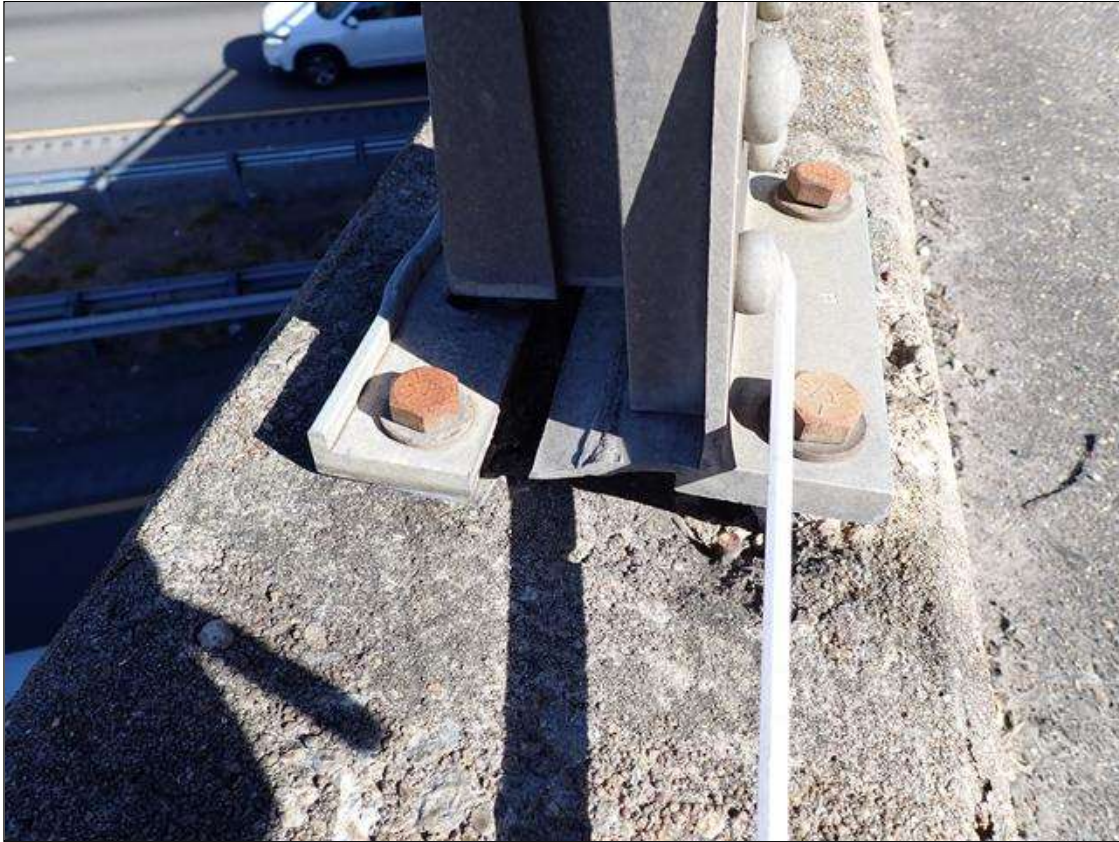
Span 2 Left Bridge Rail: (PAR) impact damage to left bridge rail at 3rd vertical post from bent 1. base plate is broken off along the weld and spalls under the base plate with two of four anchor bolts exposed. impact damage is above eastbound I-40 right travel lane. rail and post are intact
