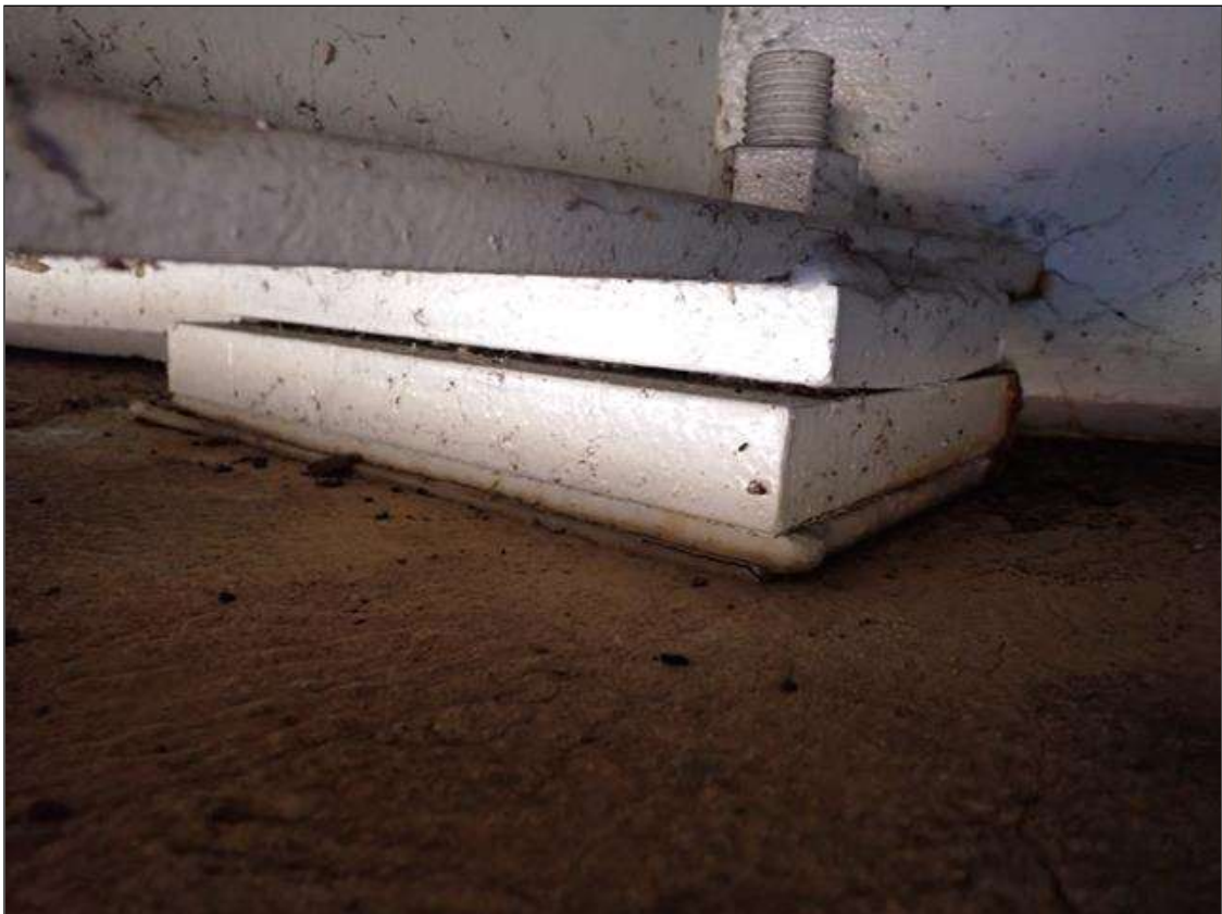
end bearing assembly
