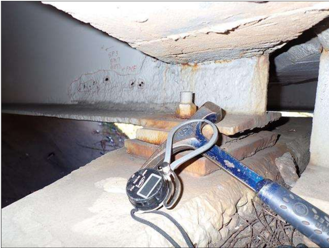
Span 4 Beam 7: (PAR) at bent 3, painted over section loss: web (1/4 inch average remaining x 8 foot x 12 inch) with corrosion holes (up to 1/4 inch diameter); bottom flange (0.45 inch average remaining x 26 inch) with corrosion reinitiated
