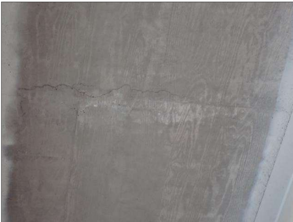
Span 1 Deck: (2) up to 2 foot wide x 12 inch long areas of delamination in deck underside, bay 3, near midspan.
