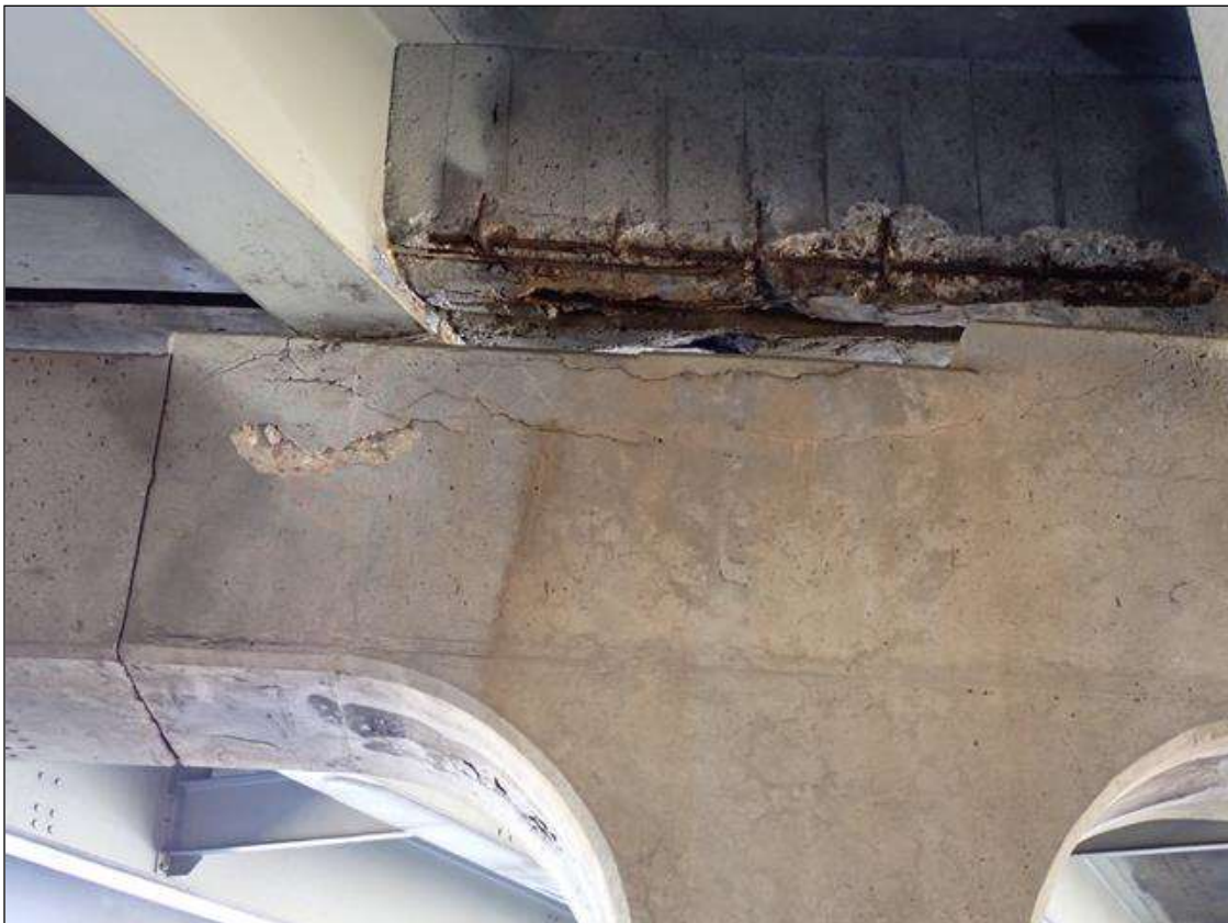
Bent 3 Cap 1: North face under bay 7, delamination 6 foot long x up to 1 foot x 4 inch x 1 inch deep in and has up to 1/8 inch wide cracks
