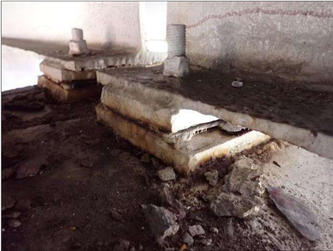
Span 3 Beam 8 - Far Bearing 8: corrosion has been arrested when painted, up to 75 percent section remaining in masonry and sole plate. west anchor bolt nut has up to 80 percent section remaining.
