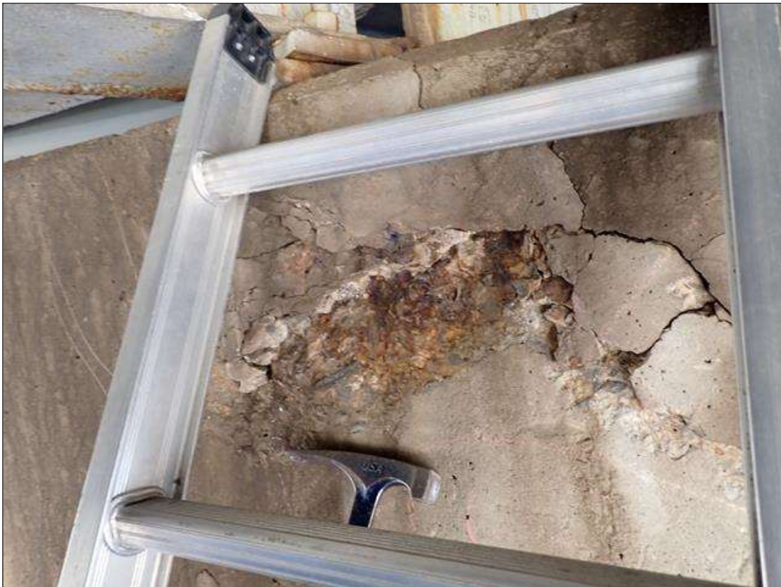
Bent 1 Cap 1: 35 inch long x 16 inch high x up to 1.5 inch deep area of delamination and spall in north face at beam 4 with exposed reinforcement. no measurable section loss.
