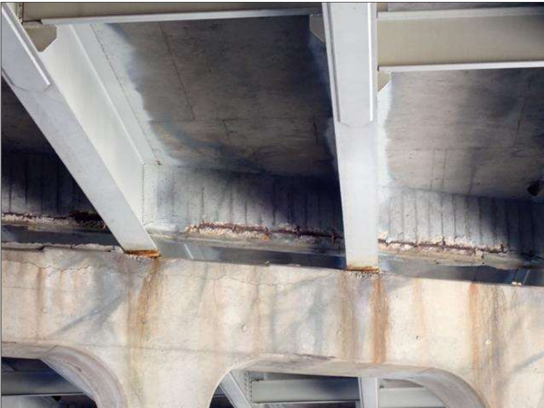
Span 3 Beam 5: (PAR) 7 foot long x up to 3 inch high x 10 inch wide area of spall in the diaphragm between beams 5 and 6 at bent 2 with exposed reinforcement. 70 percent section remaining in the exposed reinforcement.
