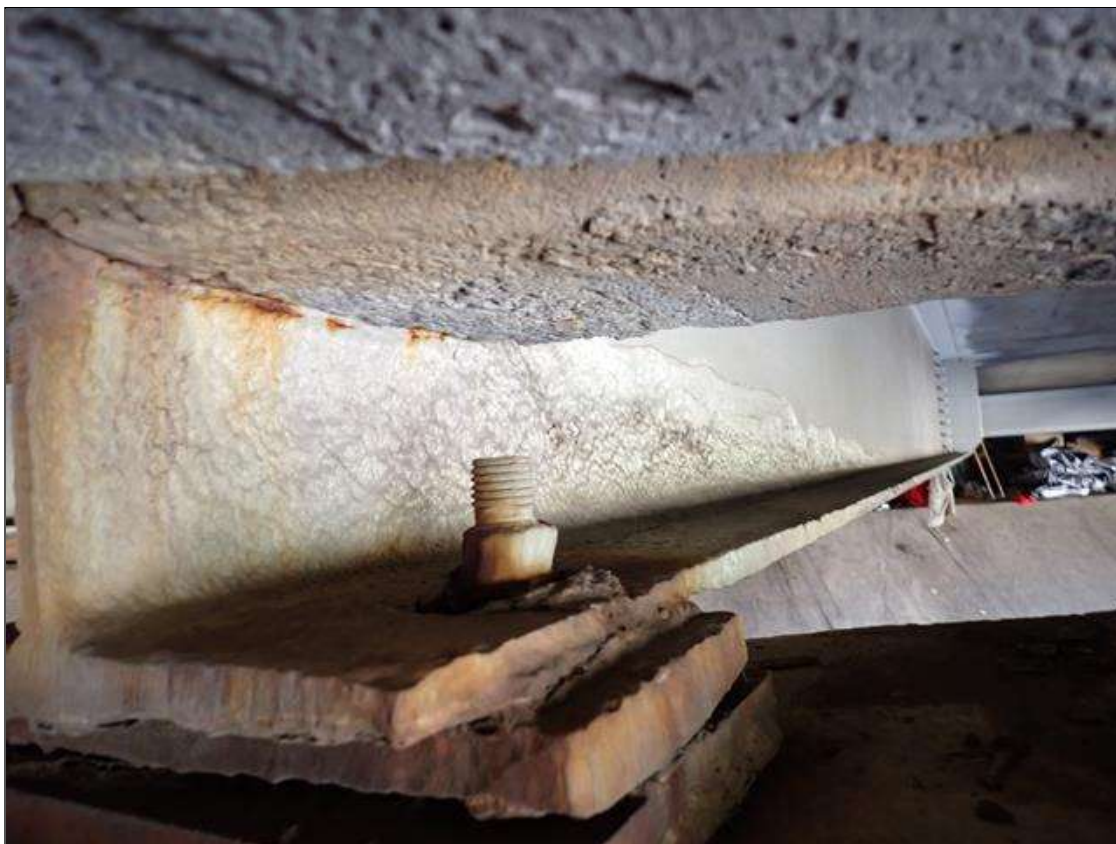
Span 4 Beam 7: (PAR) at bent 3, painted over section loss: web (1/4 inch average remaining x 8 foot x 12 inch) with corrosion holes (up to 1/4 inch diameter); bottom flange (0.45 inch average remaining x 26 inch) with corrosion reinitiated
