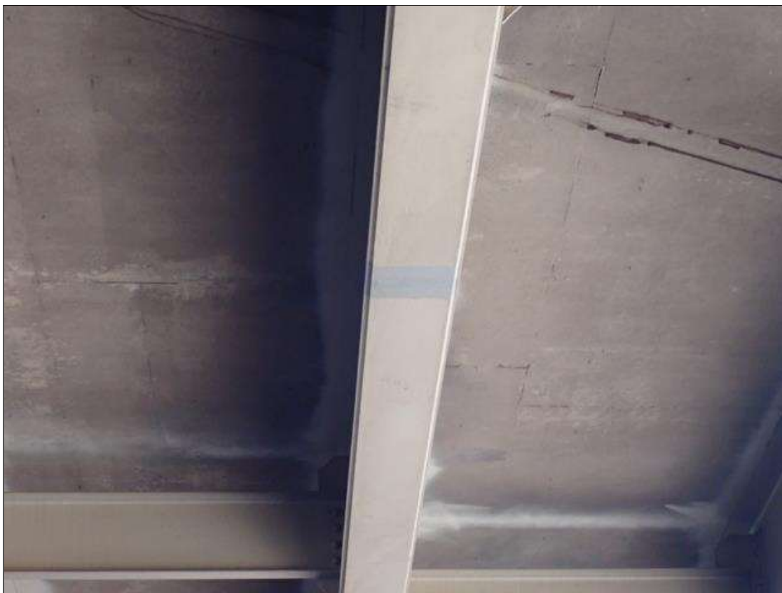
Span 3 Beam 3: 2023 new paint repair; previously noted as: SUPPLEMENTAL INSPECTION IMPACT DAMAGE 2021 :scattered scrapes
