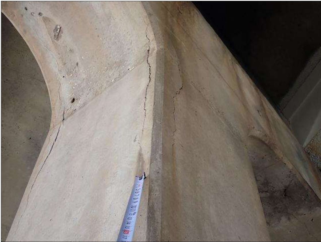
Bent 2 Pile 4: below cap, northeast and southeast corners, (2) delaminations (up to 3.5 foot x 10 inch) with cracks (1/4 inch)
