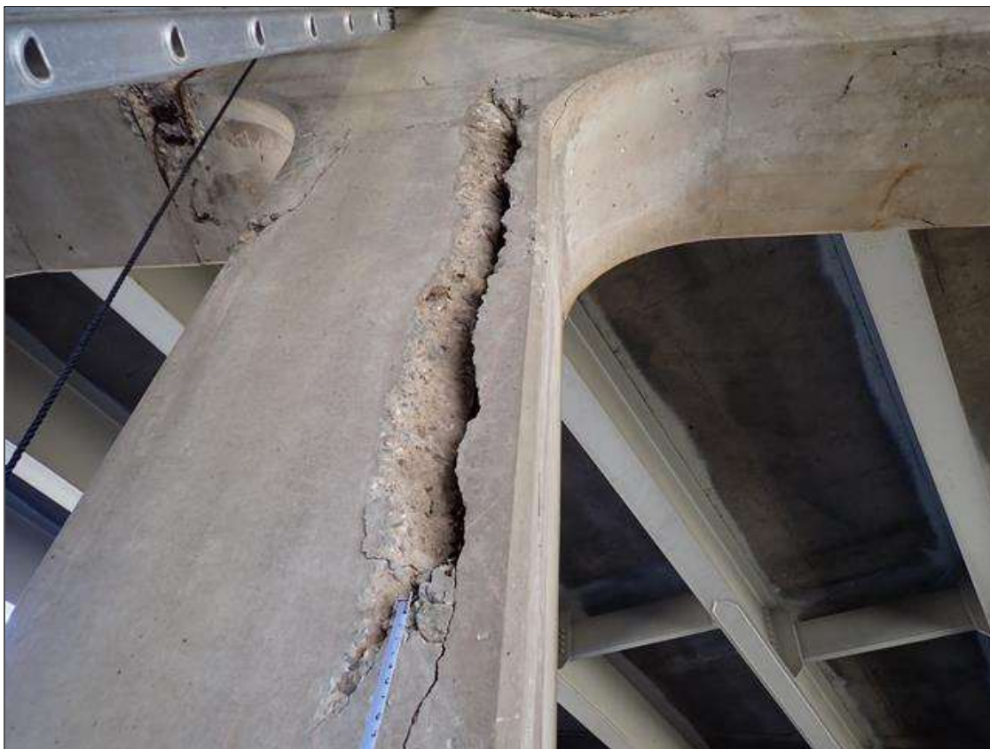
Bent 2 Pile 3: (PAR) Southeast corner 5 foot from the ground, delamination/spall [28 inch wide x 9.5 foot x up to 4 inch deep] with [1] primary exposed rusted reinforcing [75 percent remaining]
