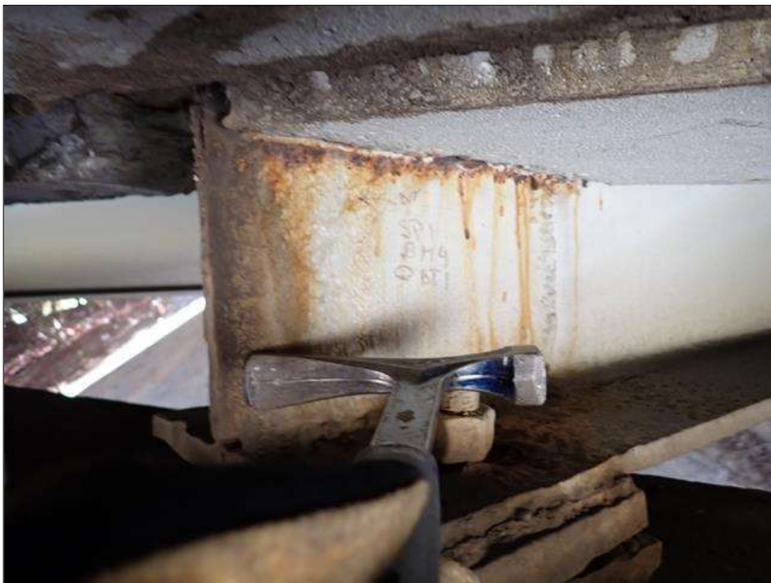
Span 1 Beam 4: at bent 1, painted over pitting up to 1/16 inch x 12 inch x 7 inch with corrosion reactivating
