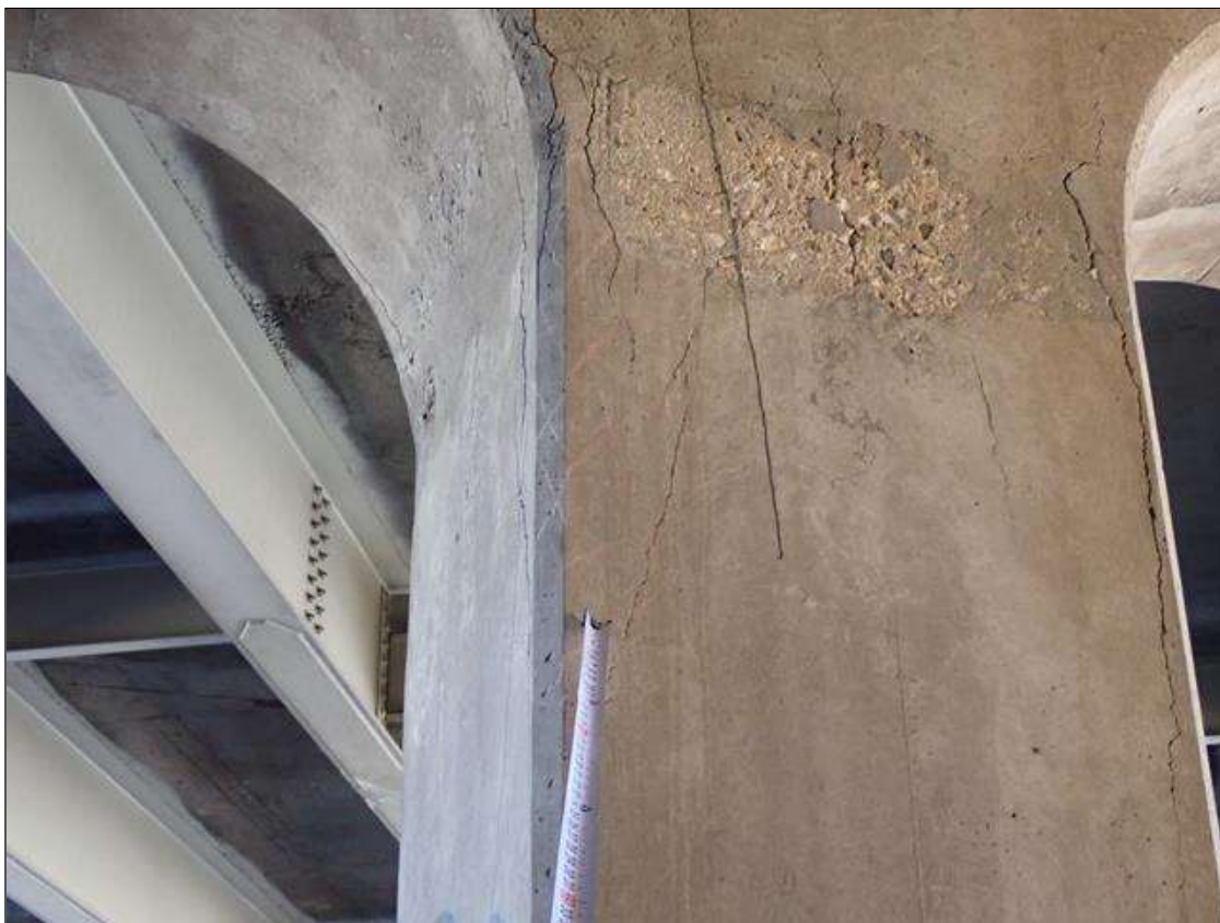
Bent 3 Pile 4: 3 foot high x 12 inch wide area of delamination and unsound concrete at northeast corner.
