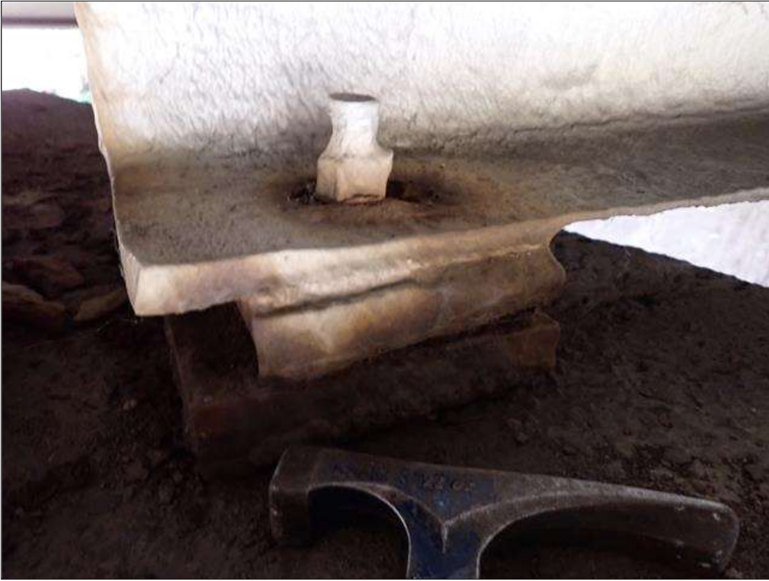
Span 1 Beam 6 - Far Bearing 6: active pack rust and section loss in masonry plate and sole plate. 80 percent section remaining. west anchor bolt nut 60 percent remaining.
