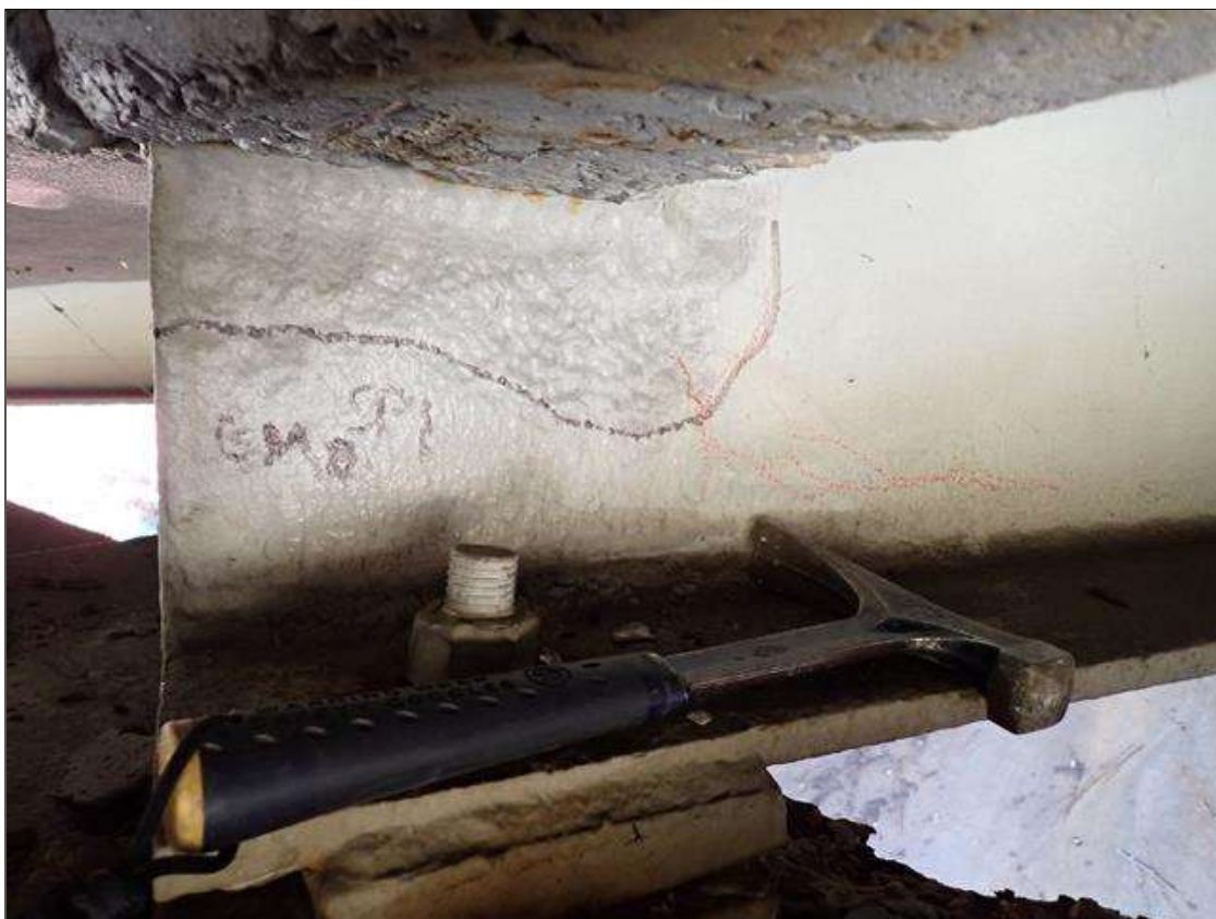
Span 1 Beam 8: (PAR) 18 inch long x up to 8 inch x 1/4 inch average remaining area of section loss in web at bent 1, spot rust present.
