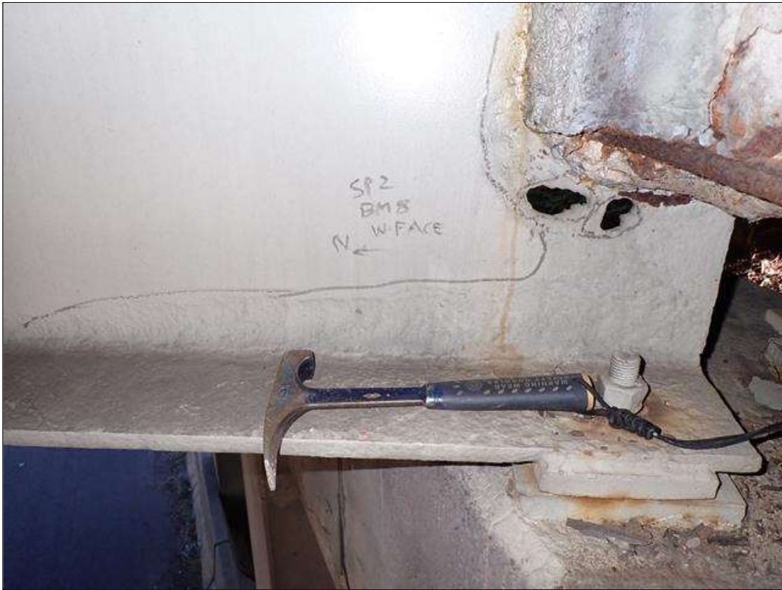
Span 2 Beam 8: (PAR) at bent 1, painted over section loss: web (1/4 inch average remaining x 24 inch x 12 inch) with corrosion hole (3 inch x 1 inch); bottom flange (0.56 inch average remaining x 12 inch) with corrosion reinitiated
