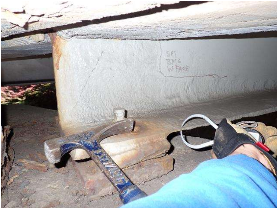
Span 1 Beam 6: (PAR) at bent 1, painted over section loss: web (1/4 inch average remaining x 3 foot x 8 inch); bottom flange (0.42 inch average remaining x 20 inch) with corrosion reinitiated
