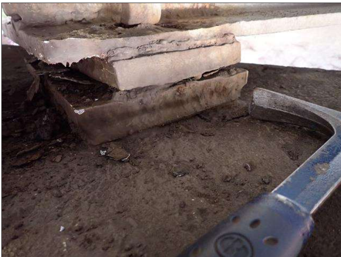
Span 1 Beam 4 - Far Bearing 4: arrested pack rust and section loss in masonry plate and sole plate. 80 percent section remaining.
