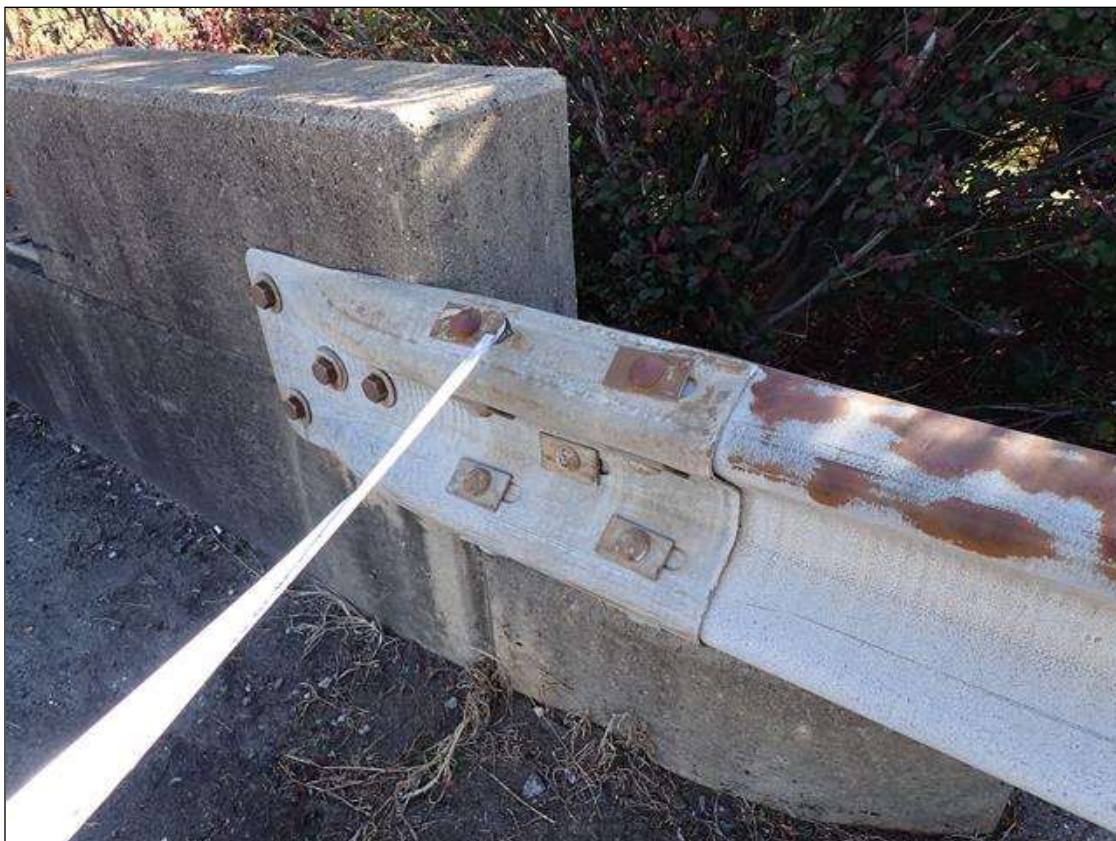
(PAR) southeast guardrail attachment, improper lap
