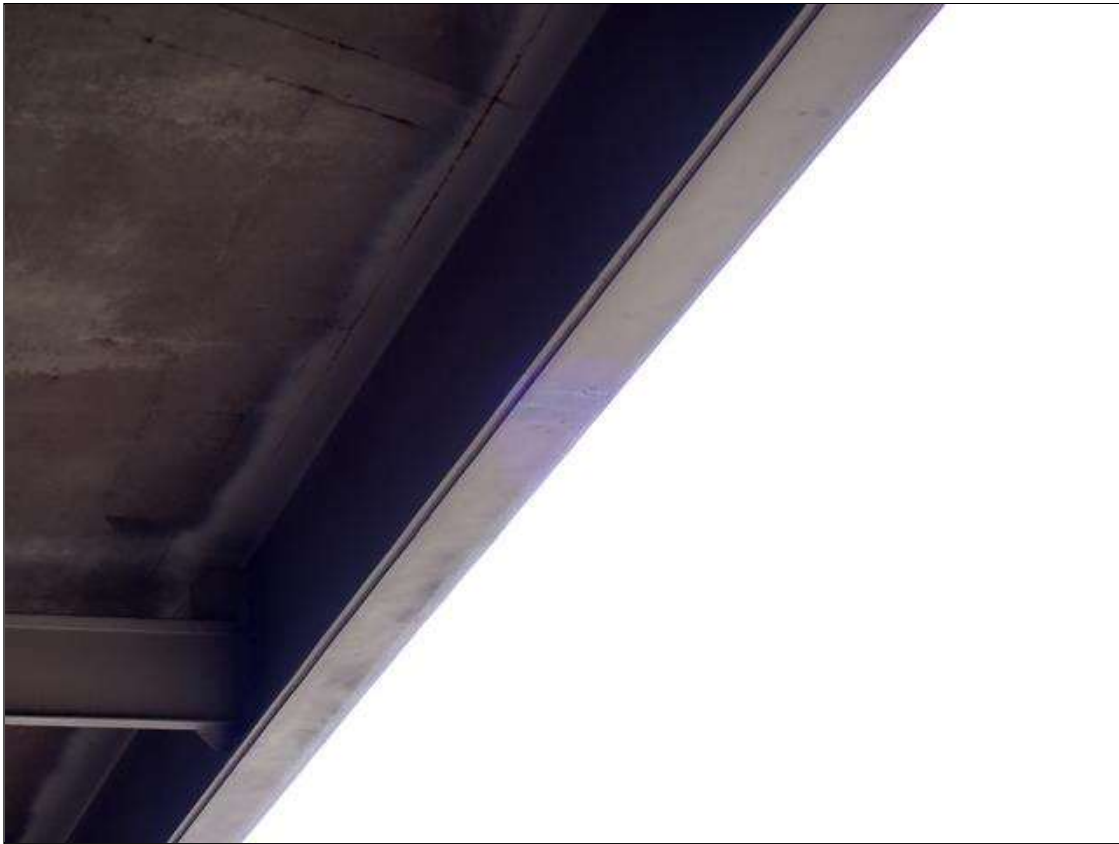
Span 3 Beam 1: (2023 no apparent change since previous inspection) SUPPLEMENTAL INSPECTION IMPACT DAMAGE 2021 :scattered scrapes
