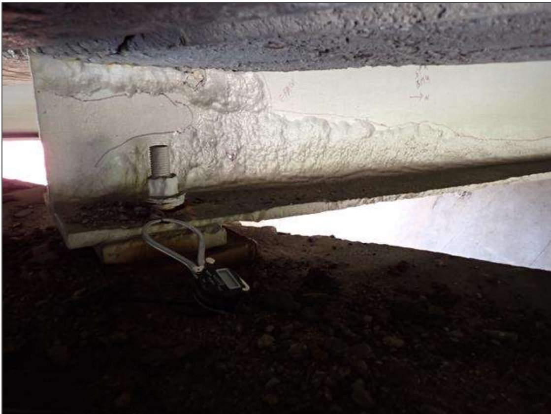
Span 4 Beam 4: (PAR) at bent 3, painted over section loss: web (1/4 inch average remaining x 5.5 foot x 10 inch) with corrosion holes (up to 1 inch x 1/2 inch); bottom flange (0.45 inch average remaining x 4 foot)
