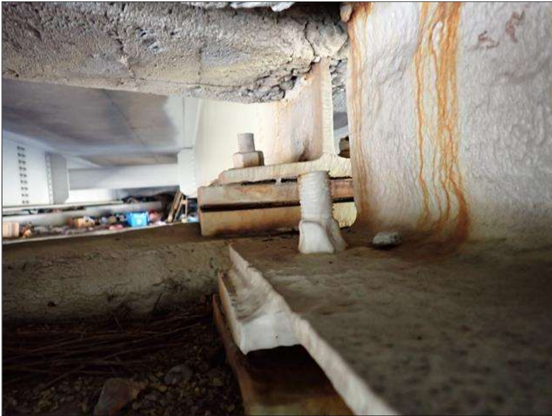
Span 3 Beam 6 - Far Bearing 6: corrosion has been arrested when painted, 75 percent section remaining in masonry and sole plate. west anchor bolt nut has 20 percent section remaining
