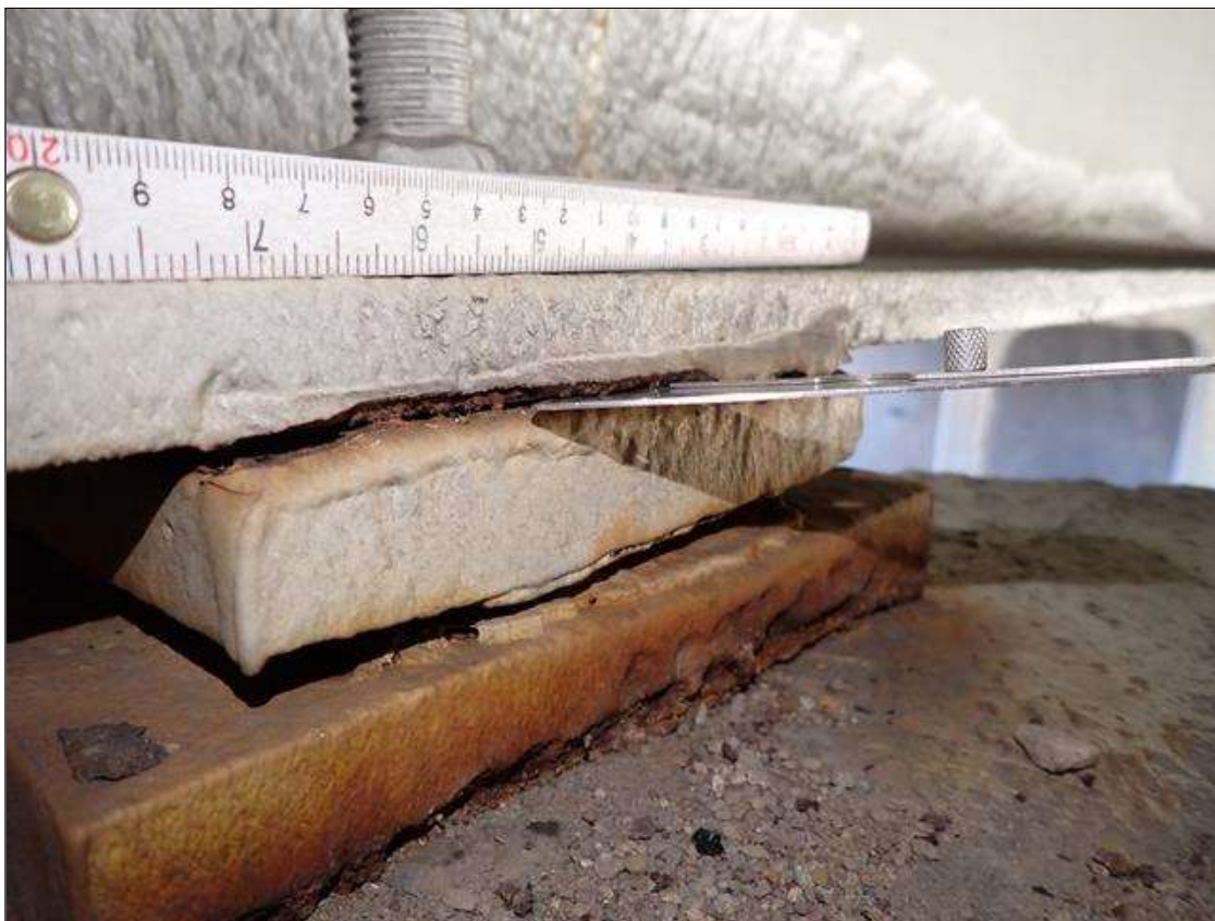
Span 3 Near Bearing 7: (PAR) east weld between sole and bottom flange, broken
