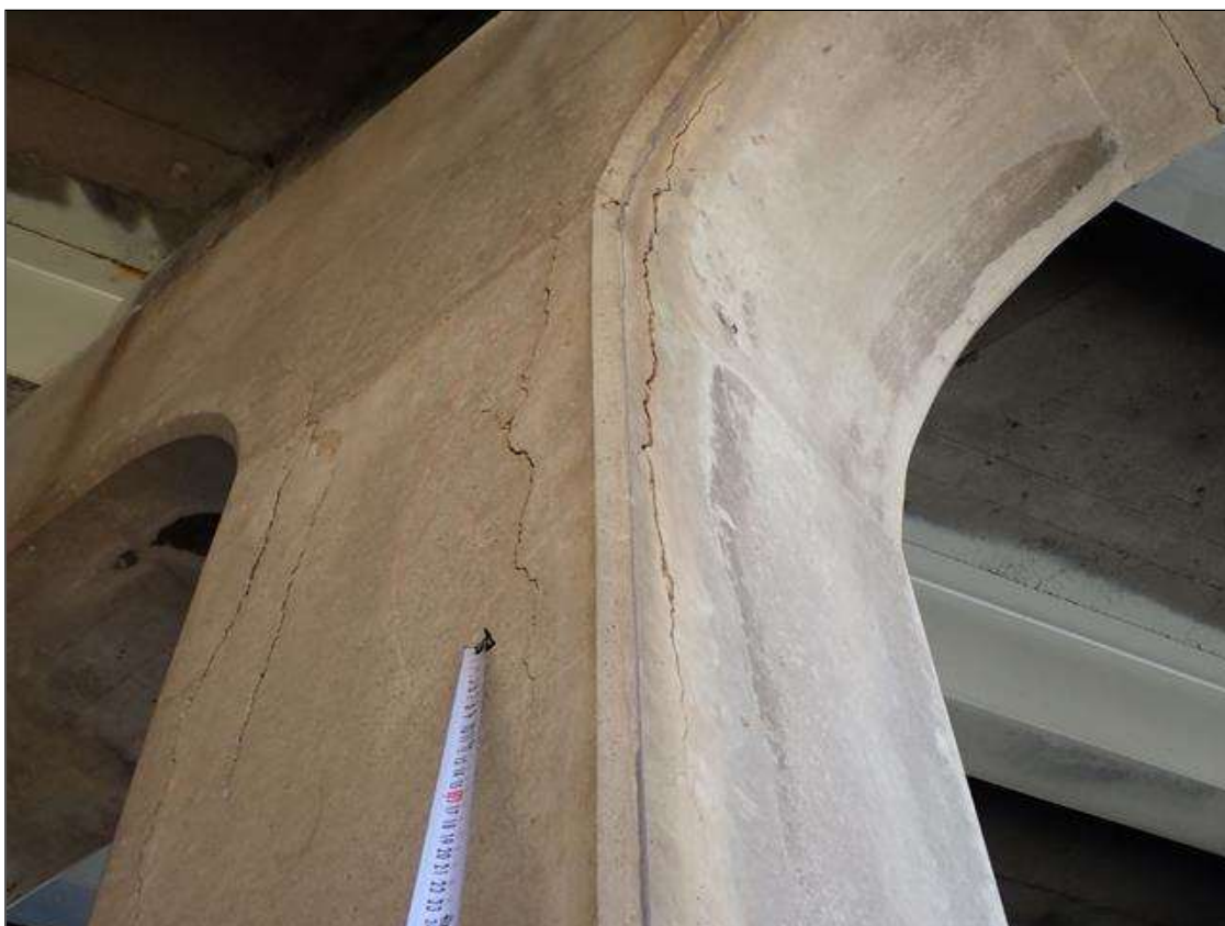
Bent 3 Pile 3: 4 foot high x 12 inch wide area of delamination and unsound concrete in north face. similar condition in west face.
