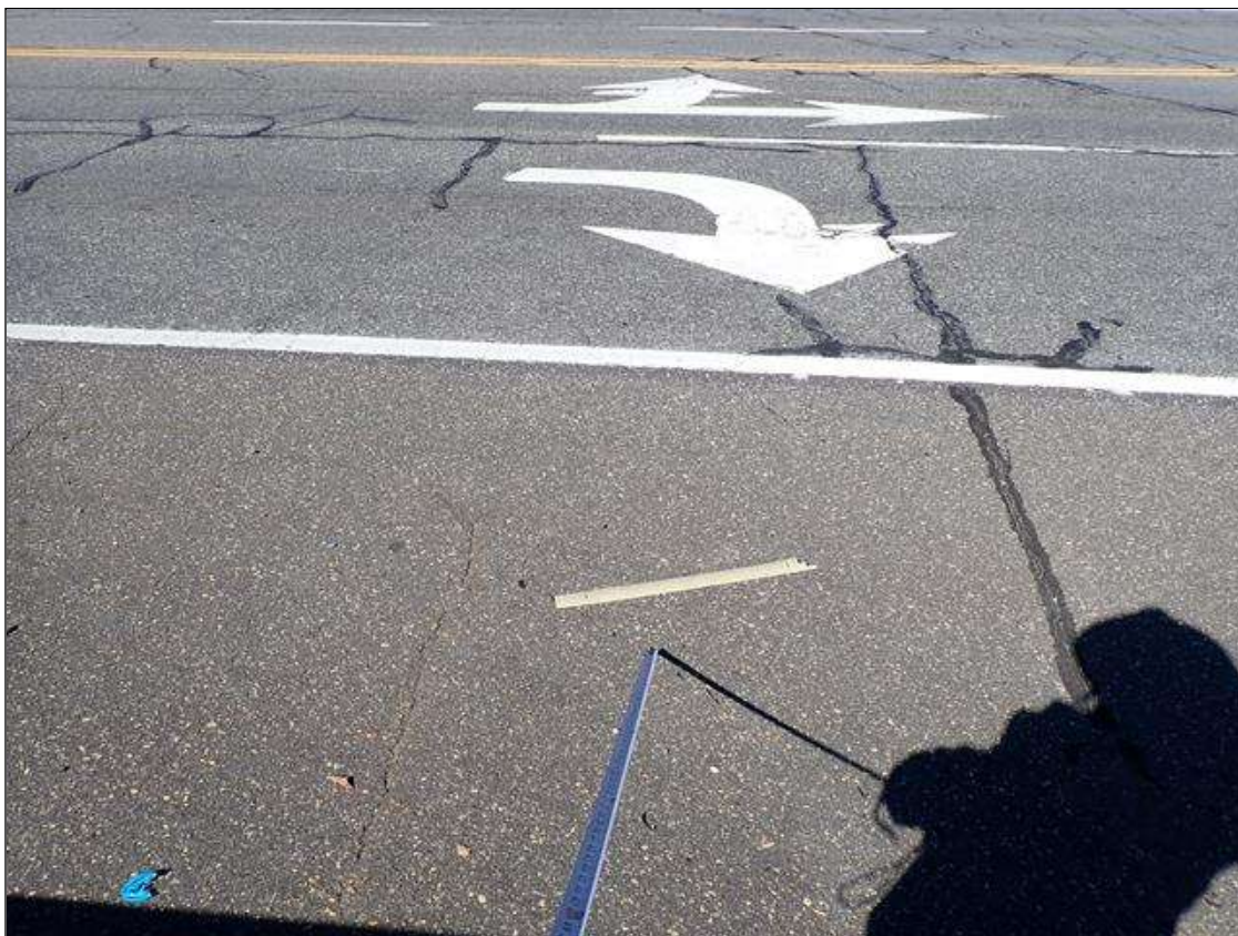
Span 4 Wearing Surface: throughout asphalt wearing surface, partially sealed transverse and longitudinal cracks (up to 1/8 inch x 40 foot)
