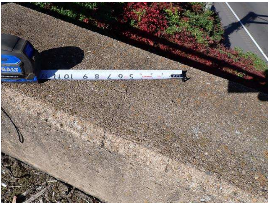
Span 1 Left Bridge Rail: along the length of parapet, vertical cracks (up to 1/32 x full height) at random
