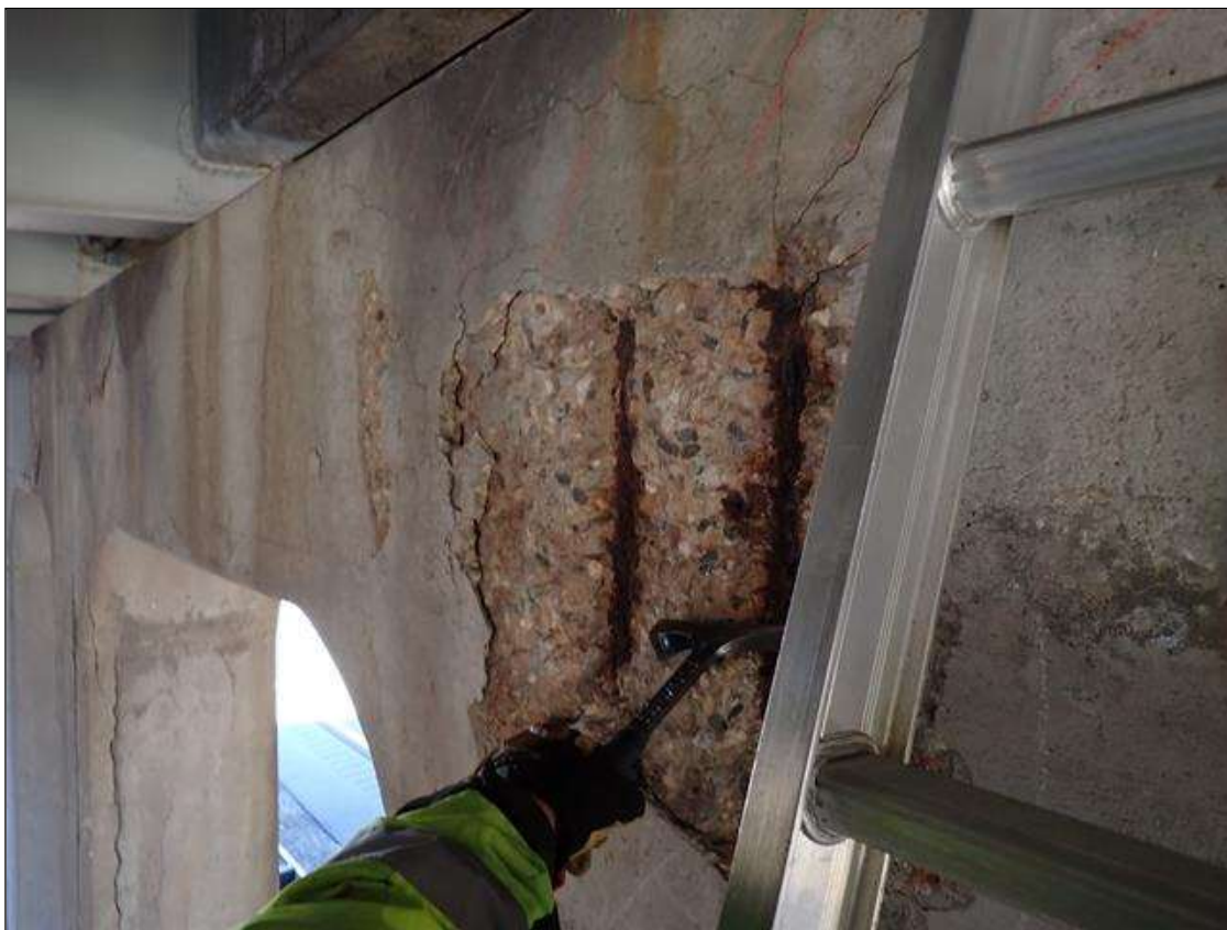
Bent 2 Cap 1: (PAR) south face, in bay 6, spall/delamination (8 foot x 4 foot x 1.5 inch deep) with exposed rusted rebar (approximately 75 percent remaining) and cracks (up to 1/16 inch)
