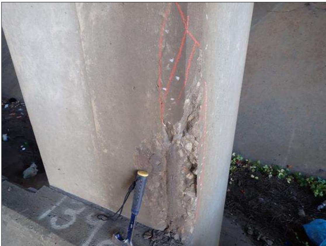
Bent 1 Pile 3: (PAR) 34 inch high x 10 inch wide x up to 2 inch deep spall with exposed rusted reinforcement.
