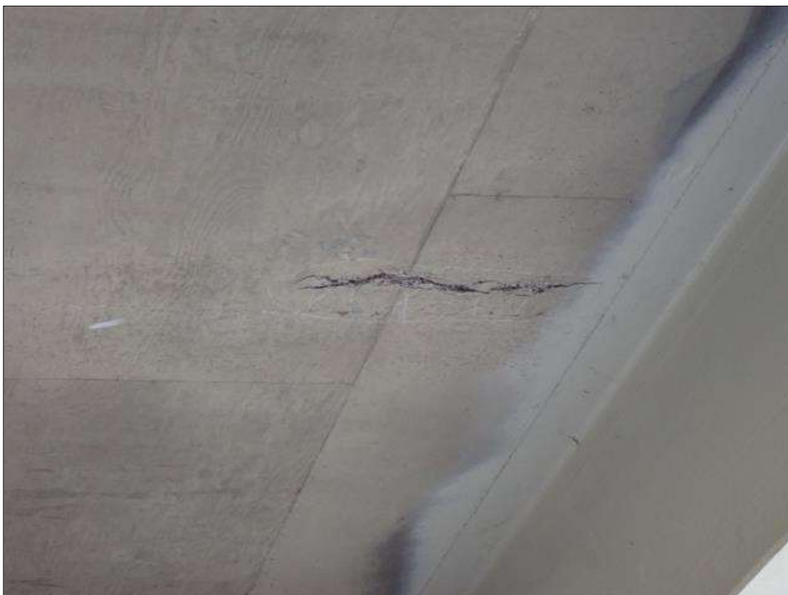
Span 4 Deck: 2 foot long x 6 inch wide x up to 1/2 inch deep area of delamination/spall in deck underside of bay 10, 15 foot from end bent 2.
