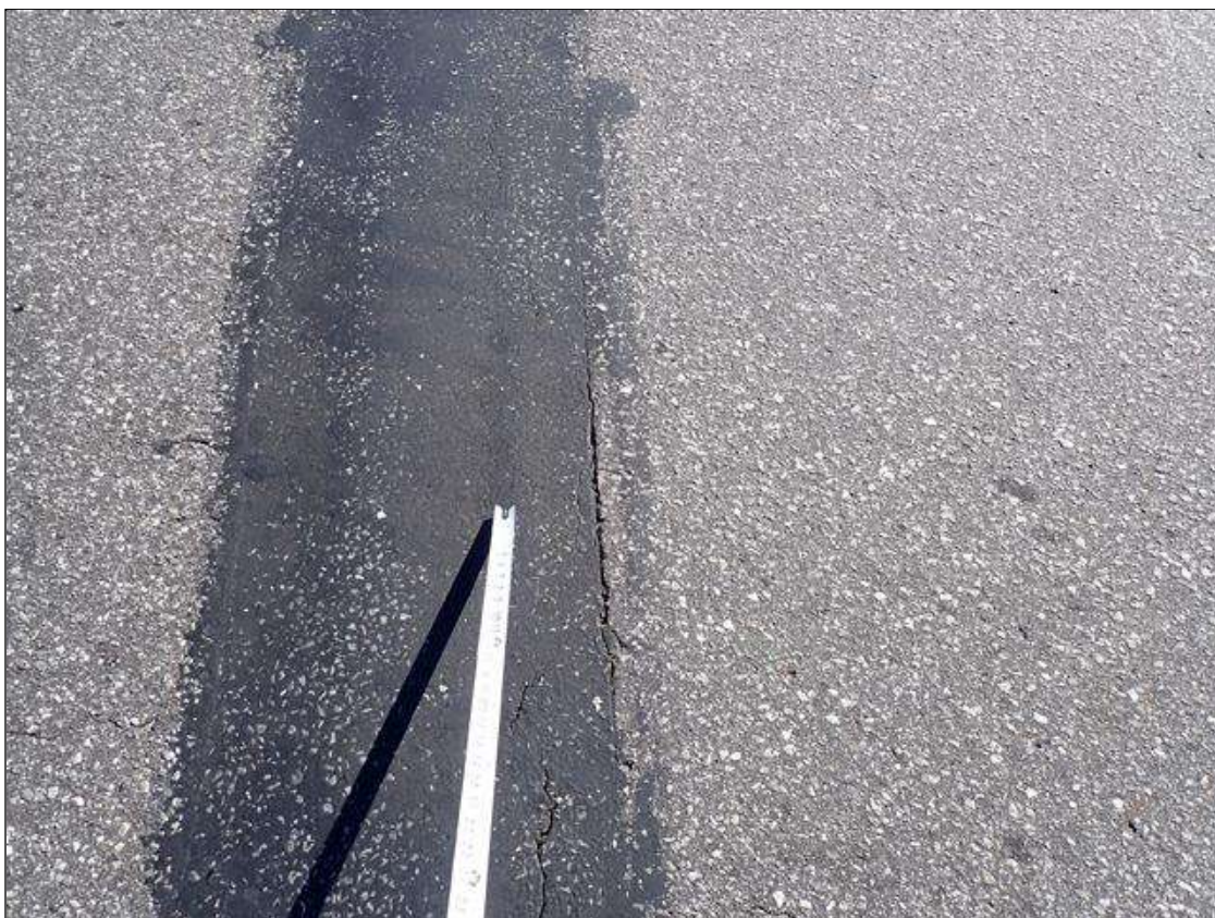
Span 3 Expansion Joint at Bent 2: along the length of the joint, adhesion loss (up to 1/8 inch wide x 2.5 foot x 3/4 inch deep) at random
