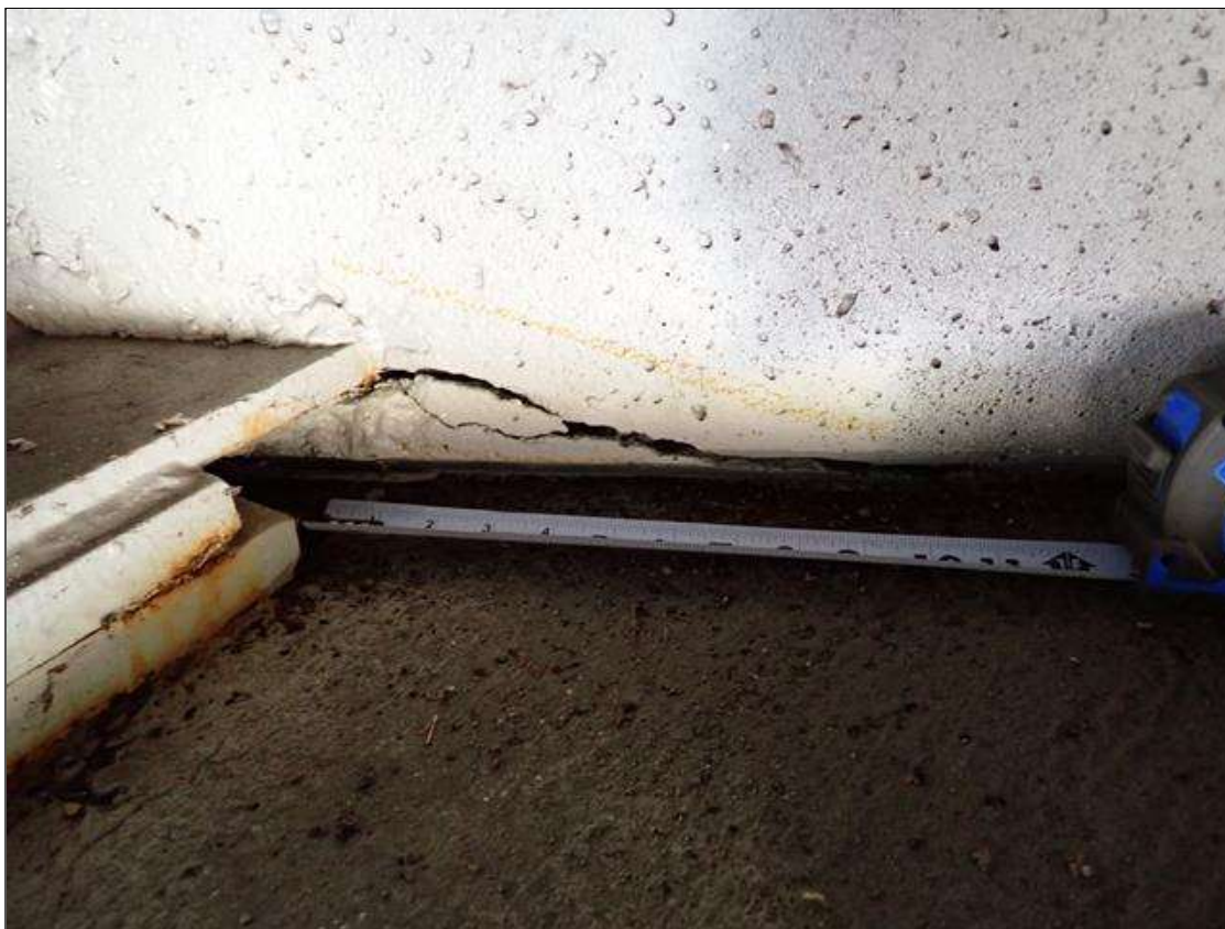
End Bent 1 Abutment: along the length of the abutment, adjacent to beam bottom flanges, spall/delaminations (up to 9 inch x 4 inch x 4 inch deep) with cracks (up to 1/8 inch)
