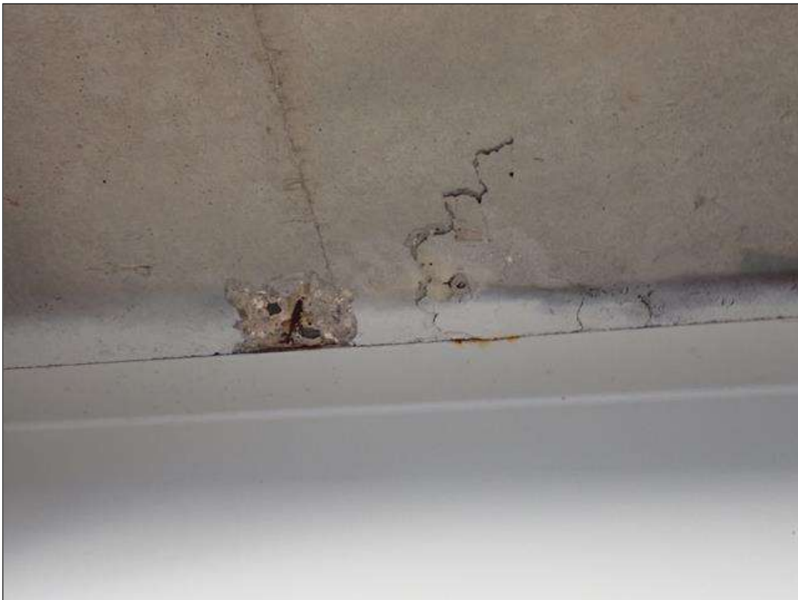
Span 1 Deck: (PAR) 6 inch diameter x 1 inch deep spall with exposed reinforcement. no measurable section loss. 18 inch long x 12 inch wide area of delamination along beam 8 top flange, in bay 7, at midspan.
