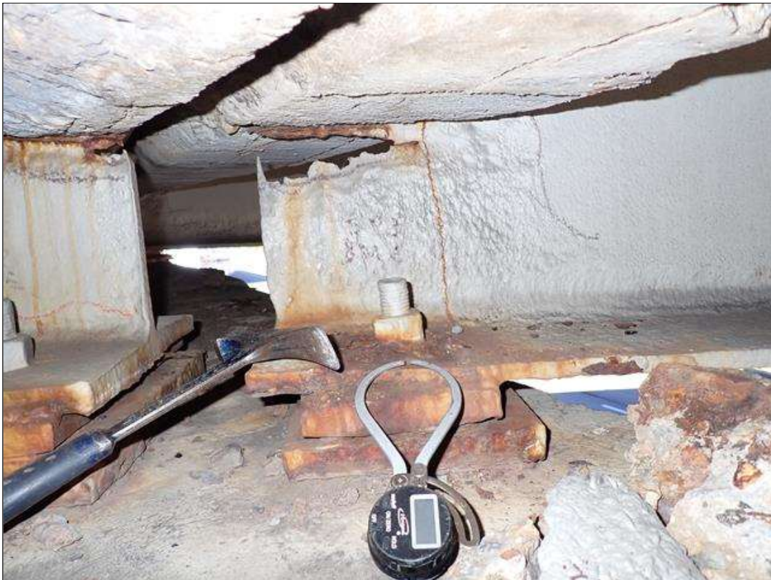
Span 3 Beam 6: (PAR) at bent 2, painted over section loss: web (1/4 inch average remaining x 3 foot x 1 foot) with corrosion hole (5 inch x 2 inch); bottom flange (0.60 inch average remaining x 2.5 foot) with corrosion reinitiated
