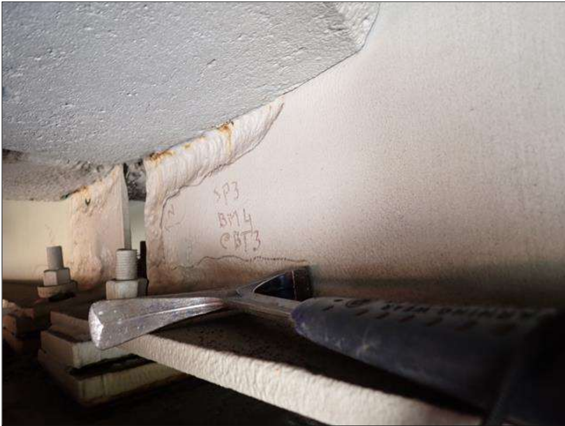
Span 3 Beam 4: (PAR) at bent 3, painted over section loss: web (1/4 inch average remaining x 15 inch x 9 inch)
