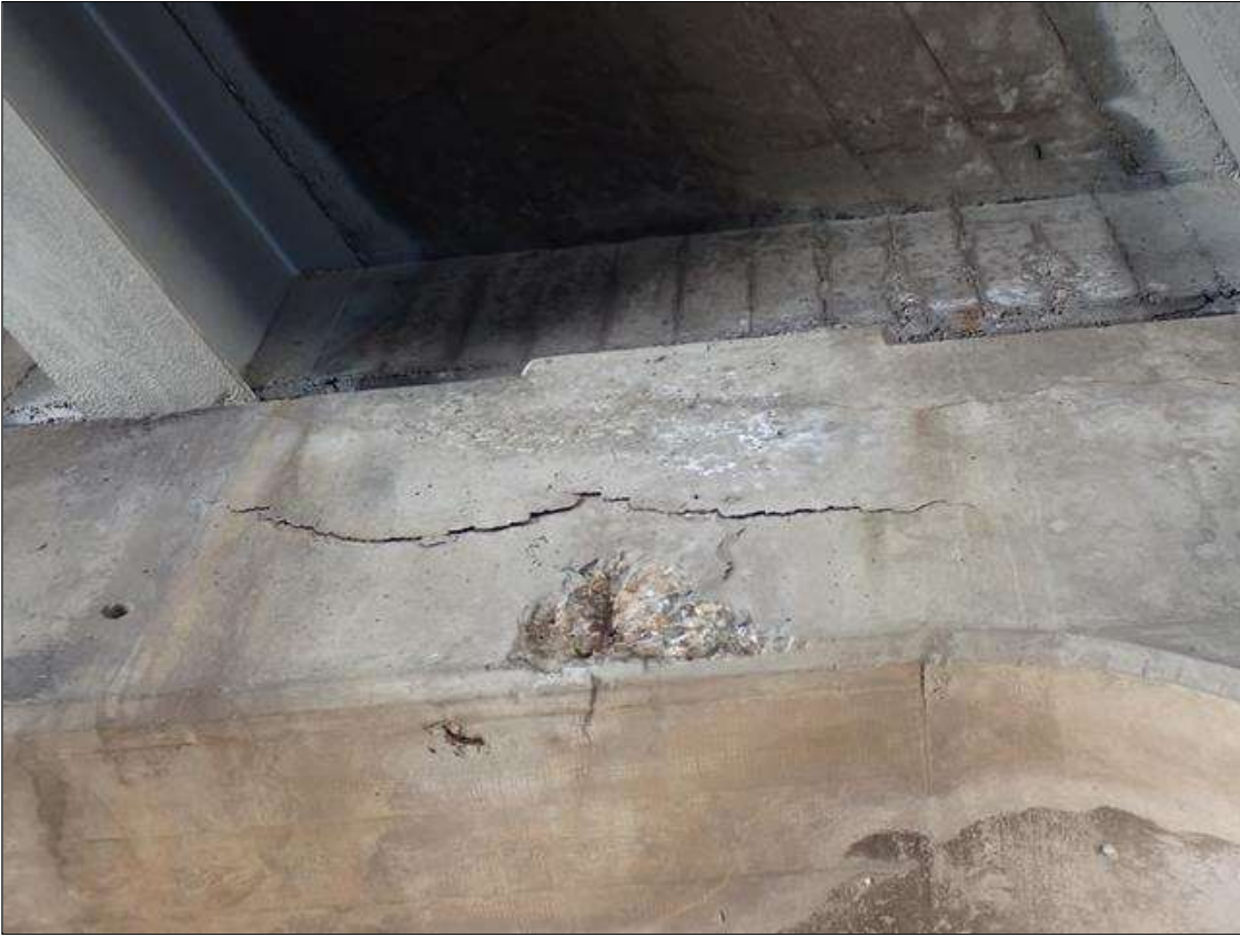
Bent 3 Cap 1: south face, in bays 4 and 5, multiple spalls/delaminations (up to 5 foot x 2 foot x 1.5 inch deep) with exposed rusted rebar
