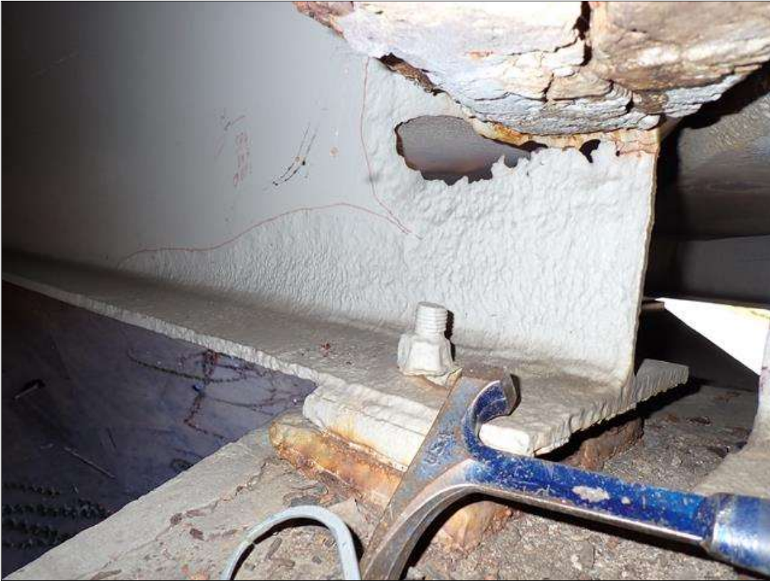
Span 4 Beam 8: (PAR) at bent 3, painted over section loss: web (1/4 inch average remaining x 34 inch x 12 inch) with corrosion hole (10 inch x 3 inch); bottom flange (0.50 inch average remaining x 34 inch) with corrosion reinitiated
