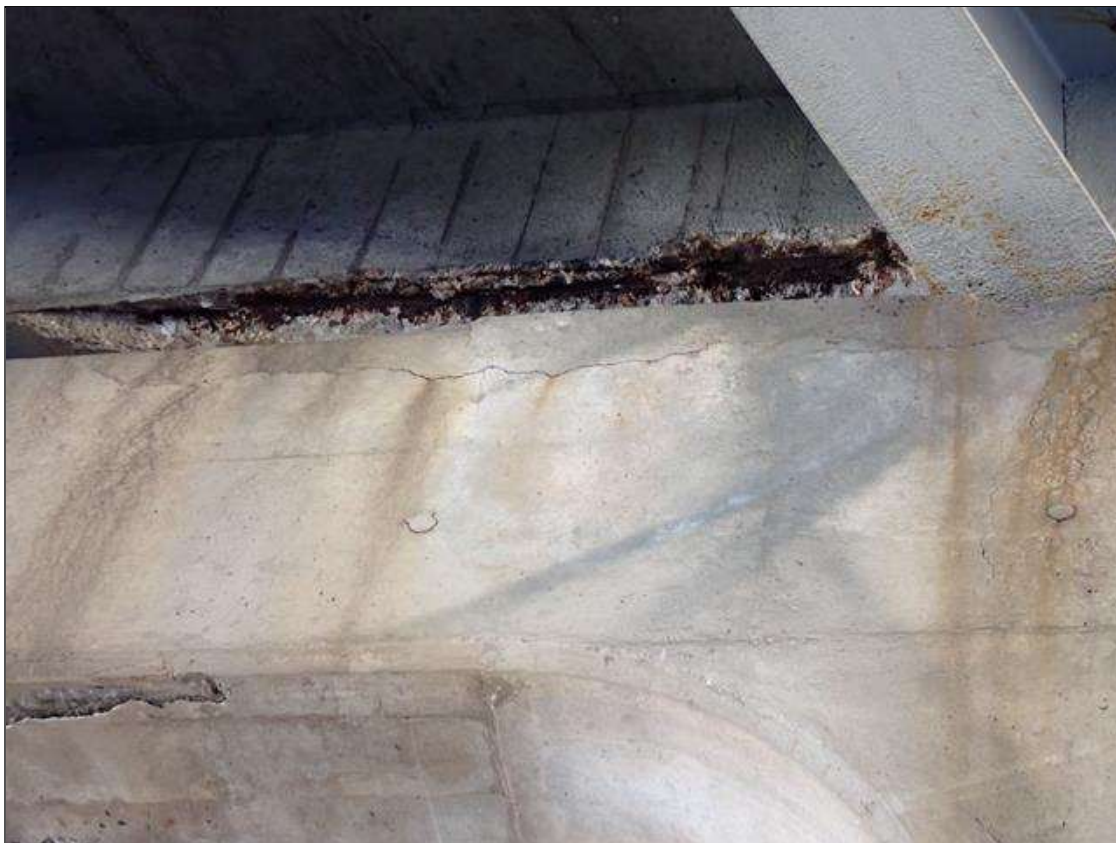
Bent 2 Cap 1: 10 foot x 1/16 inch horizontal crack in north face of cap under bays 5 and 6
