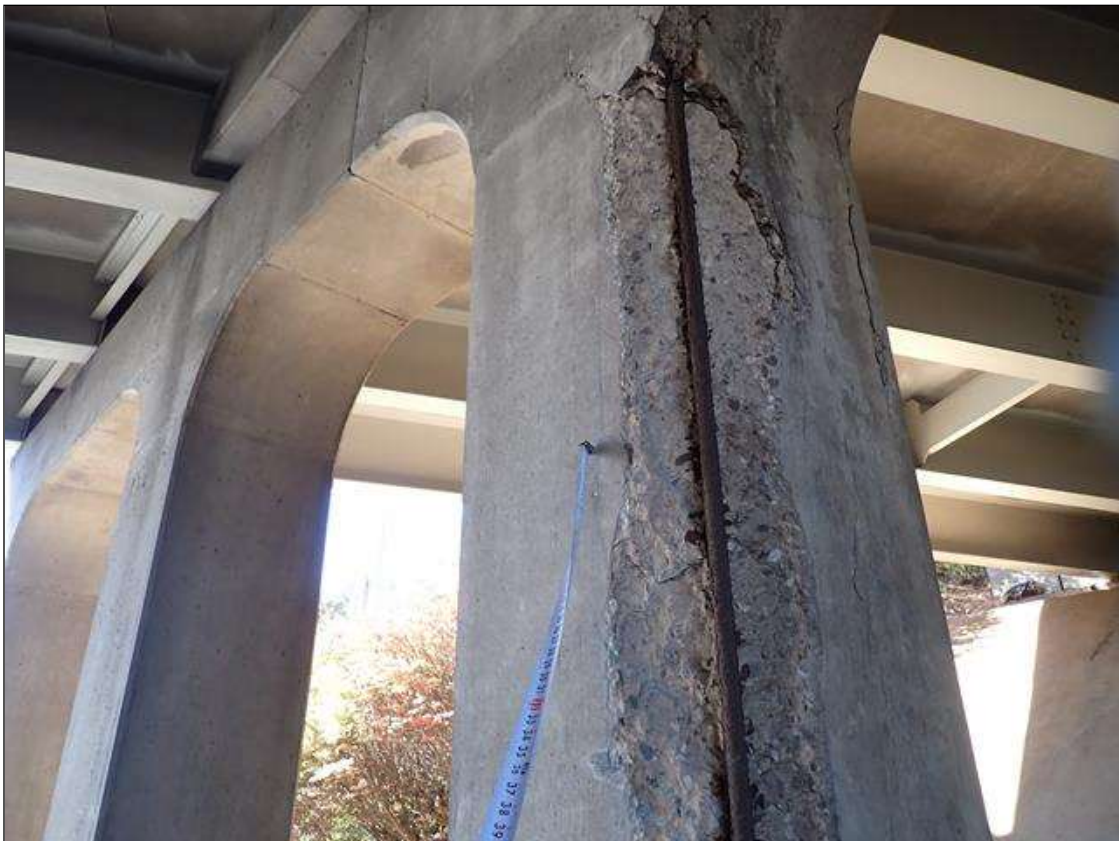
Bent 3 Pile 3: (PAR) Southeast corner above barrier rail, spall/delamination [10 foot high x up to full width x up to 4 inch deep] with primary debonded exposed rusted reinforcing 75 percent remaining
