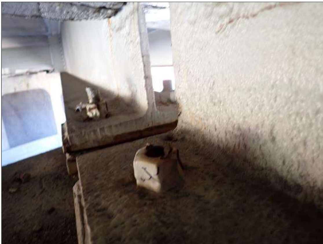
Span 2 Beam 8 - Far Bearing 8: [PAR] West face anchor bolt not visible within nut
