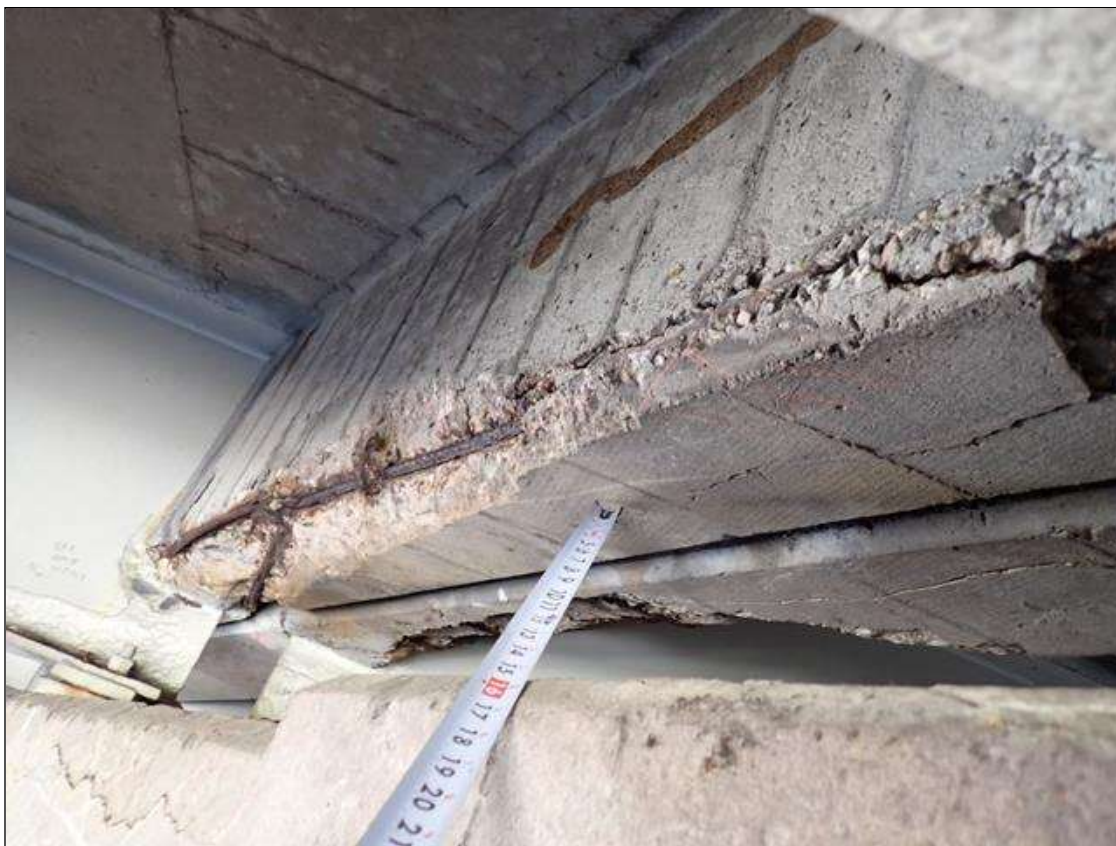
Span 2 Beam 7: (PAR) 7 foot long x 4 inch high x 4 inch wide area of spalling, delamination with the exposed reinforcement in the concrete diaphragm between beams 7 and 8 at bent 1. 70 percent section remaining in the exposed reinforcement.
