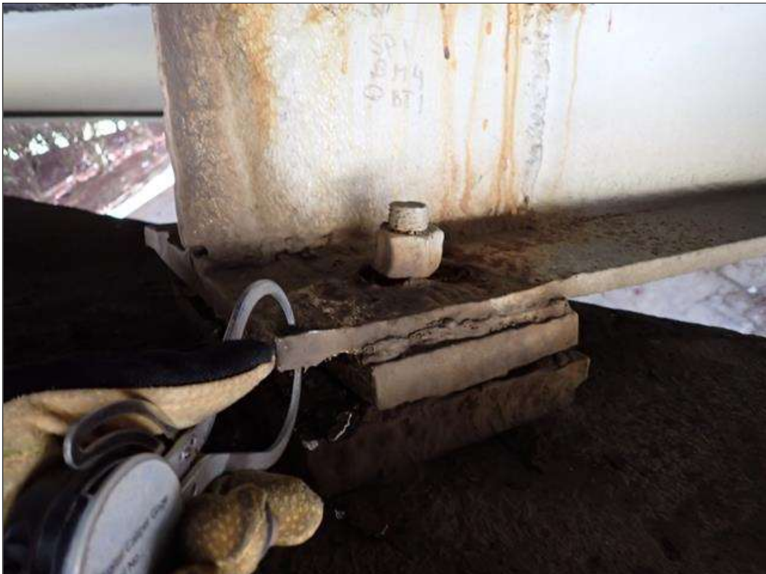
Span 1 Beam 4: (PAR) 8 inch long x full flange width x 0.55 inch remaining thickness in bottom flange with corrosion reactivating at bent 1
