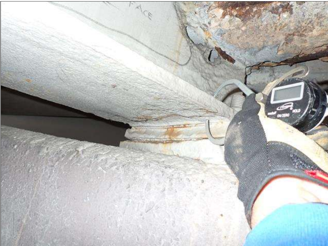
Span 2 Beam 8: (PAR) at bent 1, painted over section loss: web (1/4 inch average remaining x 24 inch x 12 inch) with corrosion hole (3 inch x 1 inch); bottom flange (0.56 inch average remaining x 12 inch) with corrosion reinitiated
