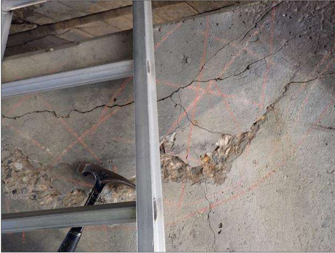
Bent 2 Cap 1: 4 foot x up to 20 inch x 1 inch deep high area of delaminated concrete in south face between beams 4 and 5.
