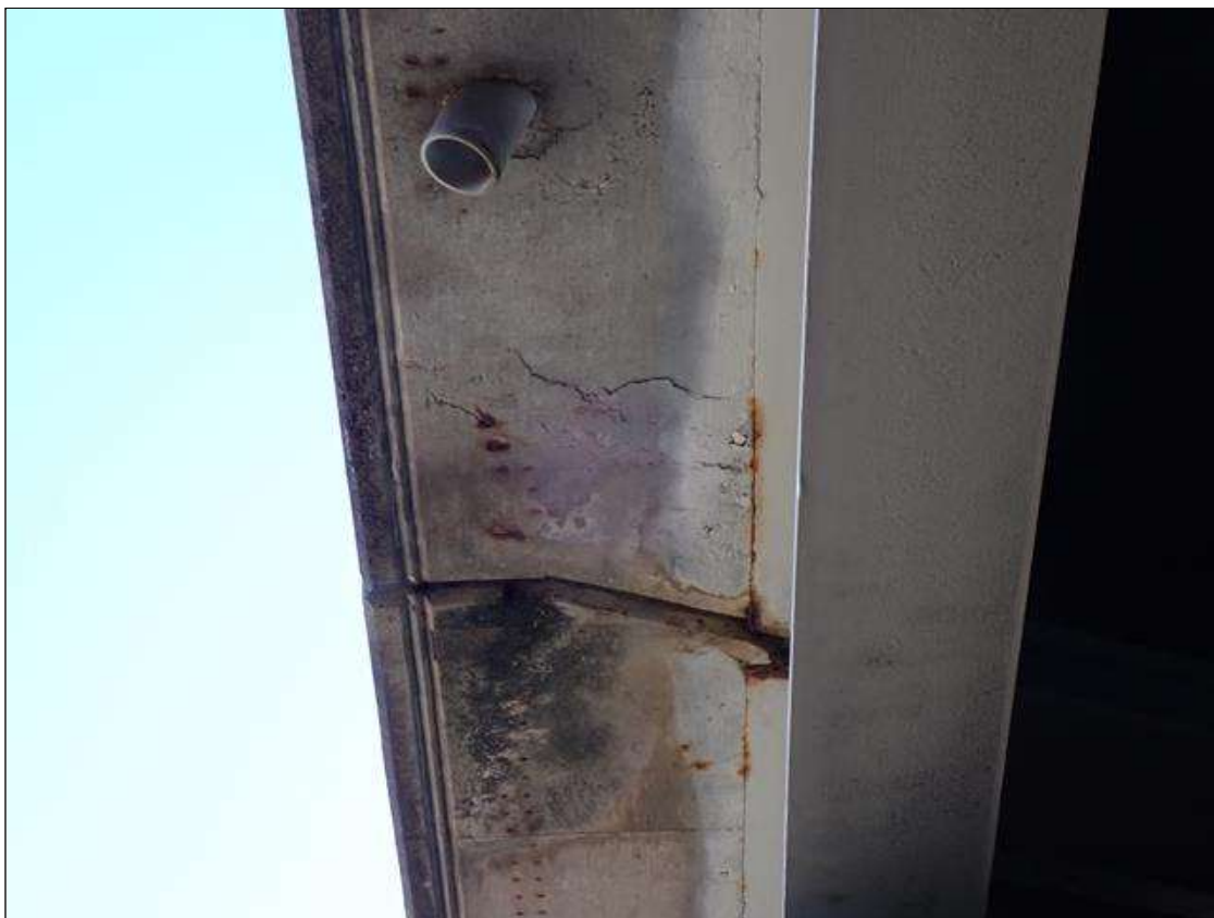
Span 1 Deck: left overhang, at bent 1, delamination (2 foot x 6 inch)
