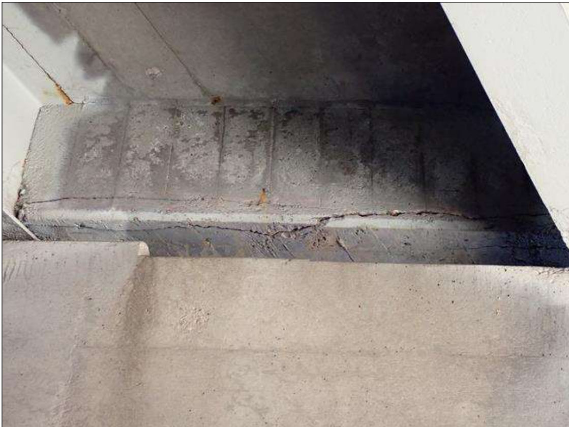
Span 4 Beam 4: 7 foot long x 8 inch wide x 4 inch along north face and 8 in along bottom face area of delamination and unsound concrete in end diaphragm at bent 3 between beams 4 and 5.
