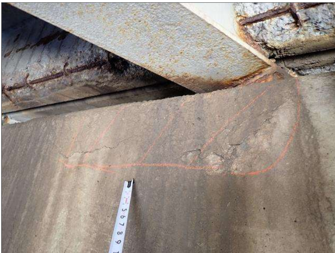
Bent 1 Cap 1: north face, below beam 5, delamination/spall [4 foot x 1 foot x 1/2 inch]
