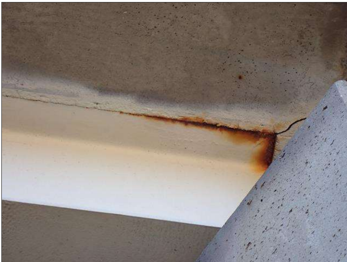
Span 3 Beam 11: at bent 3, top flange, surface rust/rust scale (1 foot)
