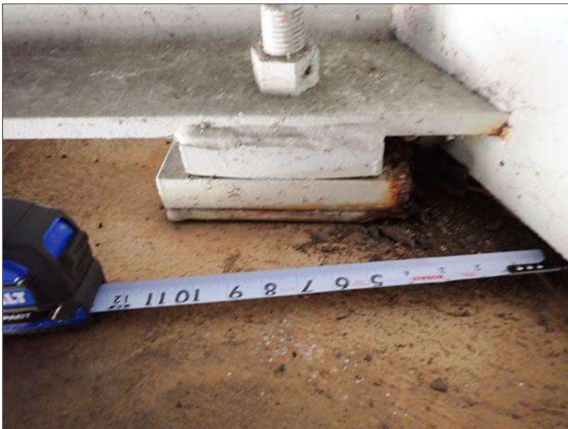
Span 1 Near Bearing 2: surface rust/rust scale
