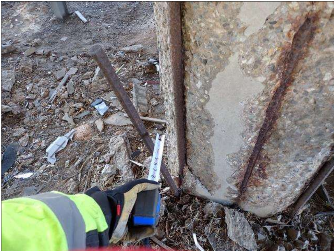
Bent 2 Pile 4: (PAR) north face, at ground, spall/delamination (full width x 7.5 foot high x 3 inch deep) extends into east and west faces (up to 7 inch) with exposed rusted and debonded rebar
