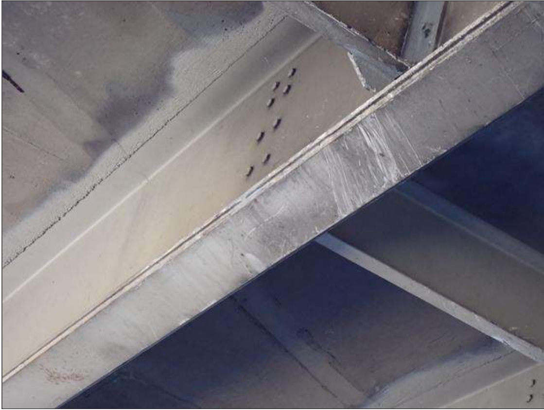
Span 3 Beam 10: (2023 no apparent change since previous inspection) SUPPLEMENTAL INSPECTION IMPACT DAMAGE 2021: 1 indentation 1 inch long x 1/2 inch deep at 18 foot-8 inch from interior. bent 3 . scattered scrapes along the web .
