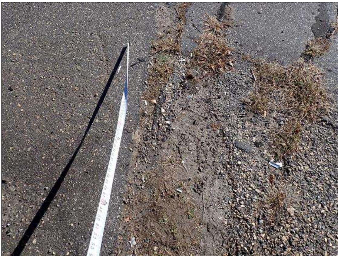
Span 1 Wearing Surface: left shoulder of asphalt over end bent 1, pothole/broken asphalt [6 foot x 8 inch x up to 1 inch deep]
