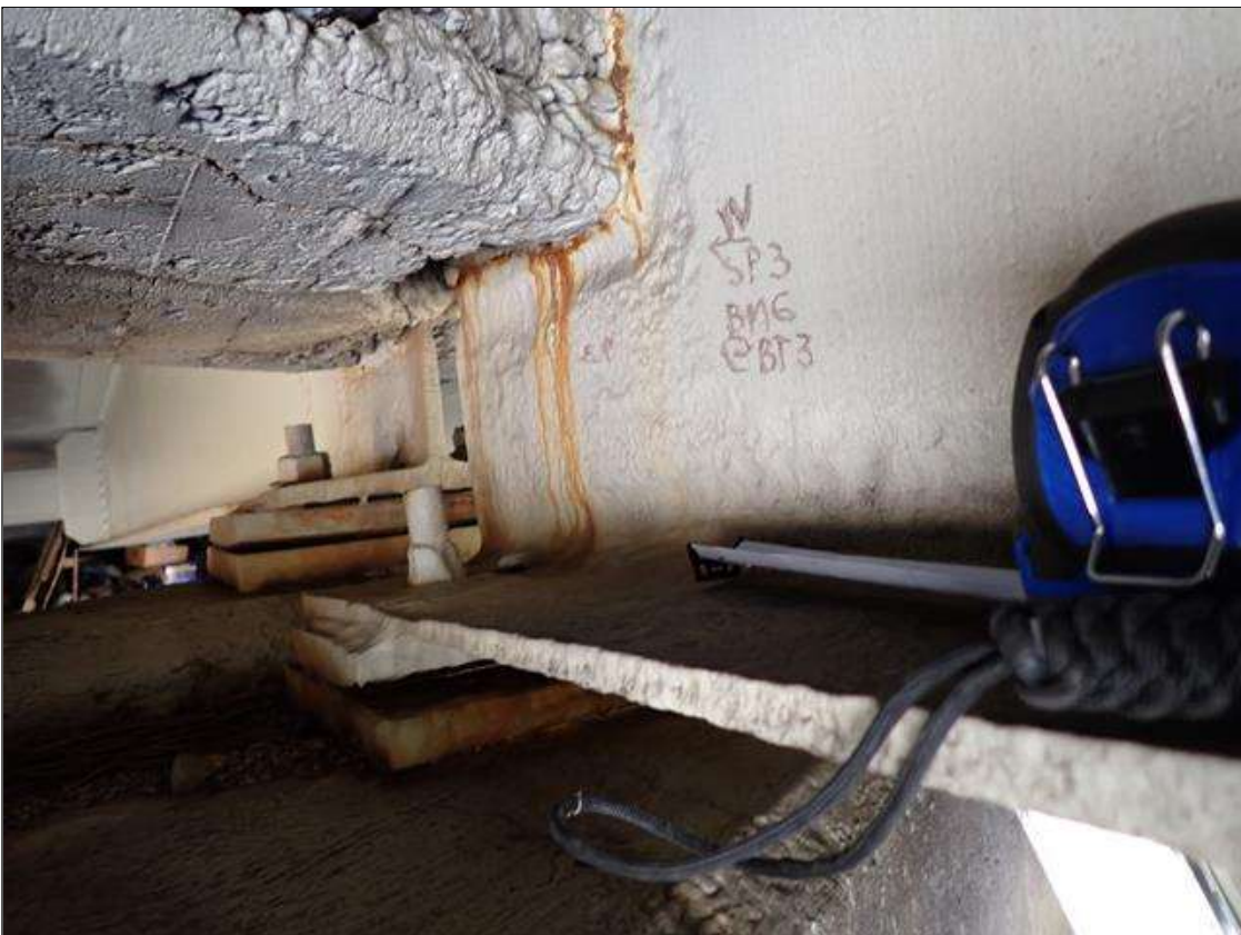
Span 3 Beam 6: (PAR) at bent 3, painted over section loss: web (1/4 inch average remaining x 20 inch x 10 inch); bottom flange (0.56 inch average remaining x 1 foot) with corrosion reinitiated
