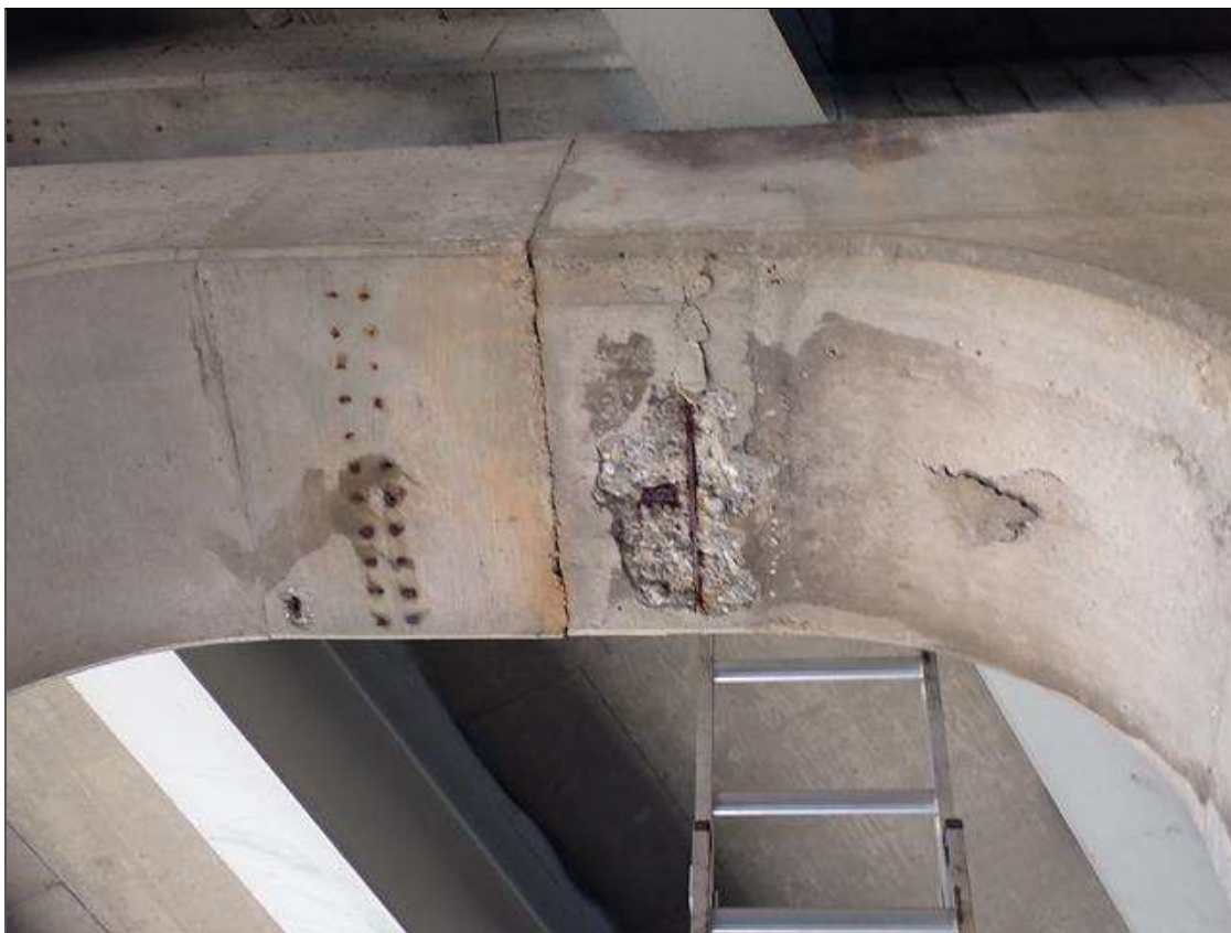
Bent 2 Cap 1: (PAR) (3) up to 1.5 foot x 1 foot wide x 1/2 inch deep spall with exposed rusted reinforcement, 80 percent remaining on underside of cap between columns 5 and 6
