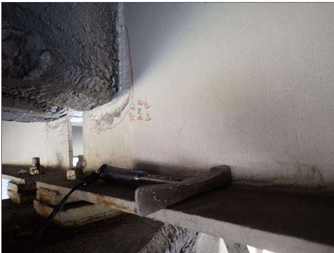
Span 2 Beam 8: (PAR) at bent 2, painted over section loss: web adjacent to diaphragm (1/4 inch average remaining x 14 inch x 8 inch); lower web (7/16 inch average remaining x 2 foot x 3 inch)
