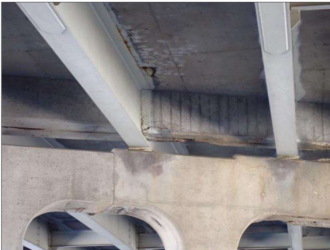
Span 3 Beam 7: multiple up to 3 foot long horizontal 1/8 inch wide cracks in end diaphragm between beams 7 and 8 at bent 2 starting at beam 8
