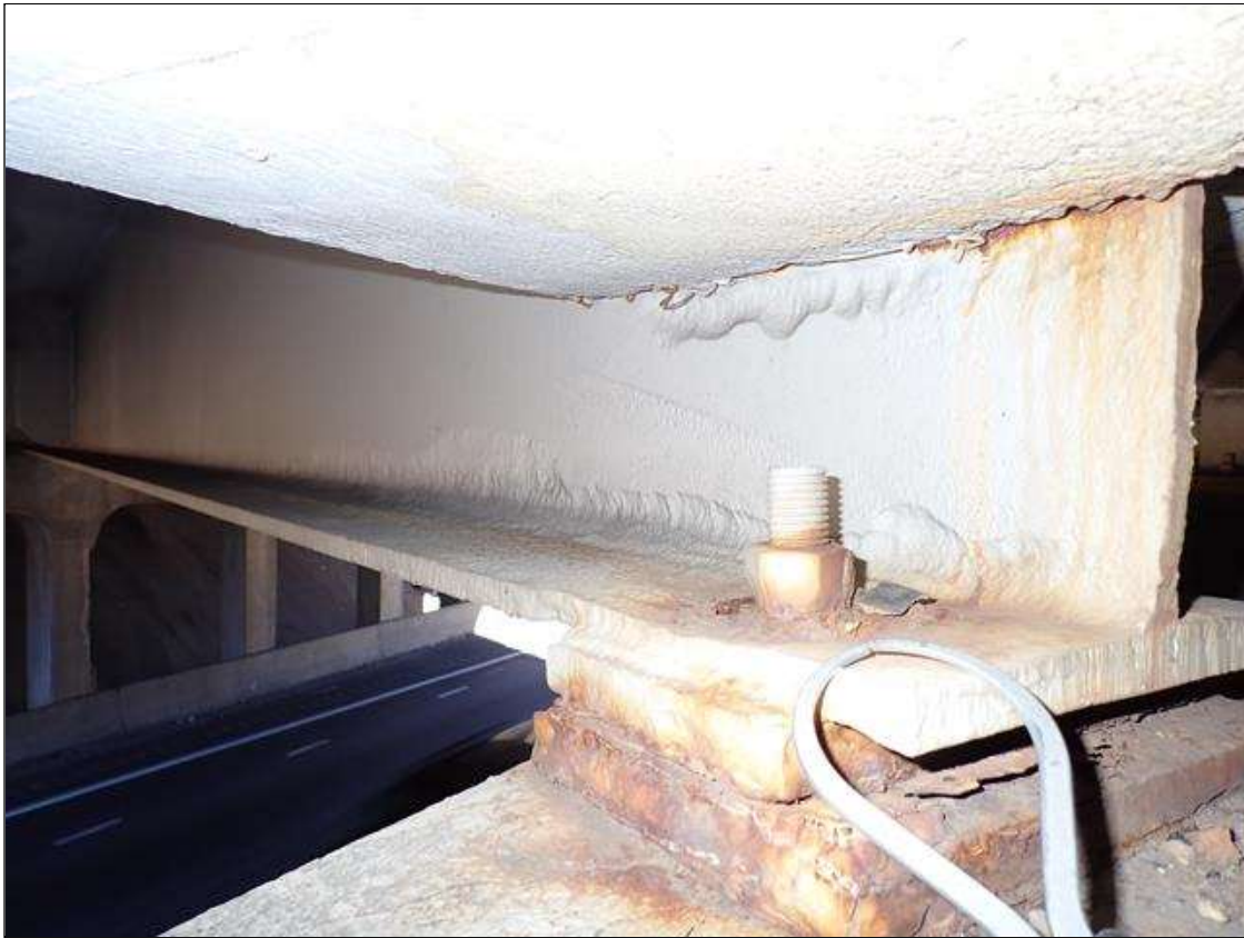
Span 3 Beam 4: (PAR) at bent 2, painted over section loss: bottom flange (0.56 inch average remaining x 9 inch), lower web (3/16 inch average remaining x 6 foot x 2 inch), web adjacent to diaphragm (3/16 inch average remaining x 12 inch x 2 inch) with corrosion reinitiated
