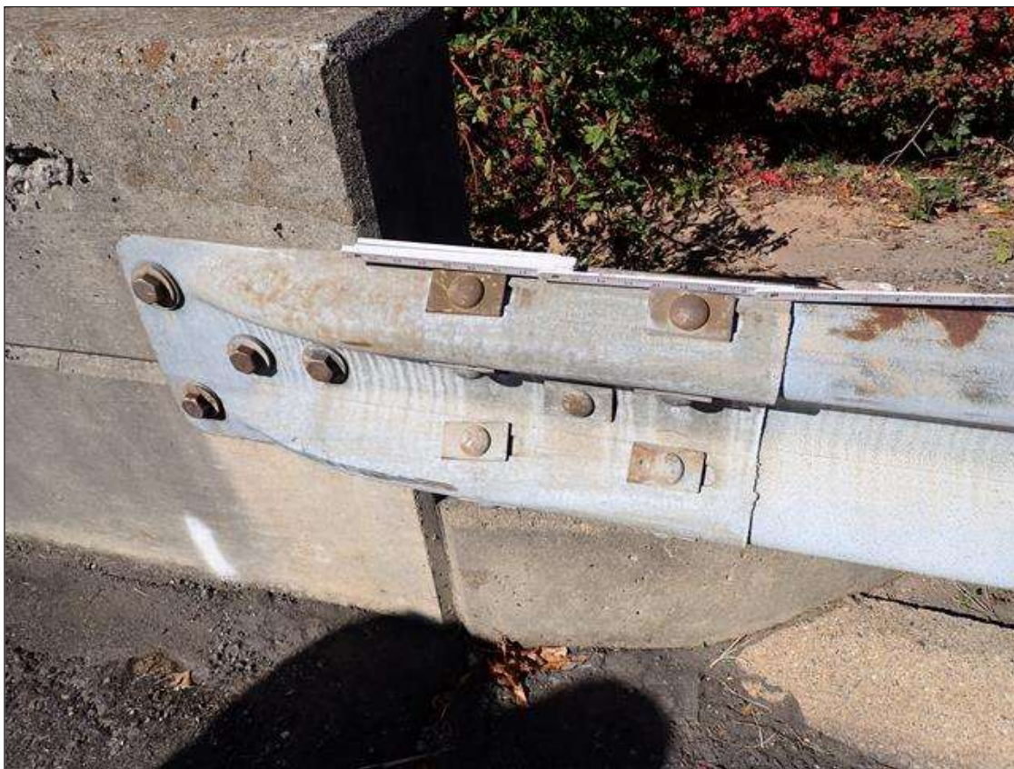
(PAR) northwest guardrail attachment, improper lap
