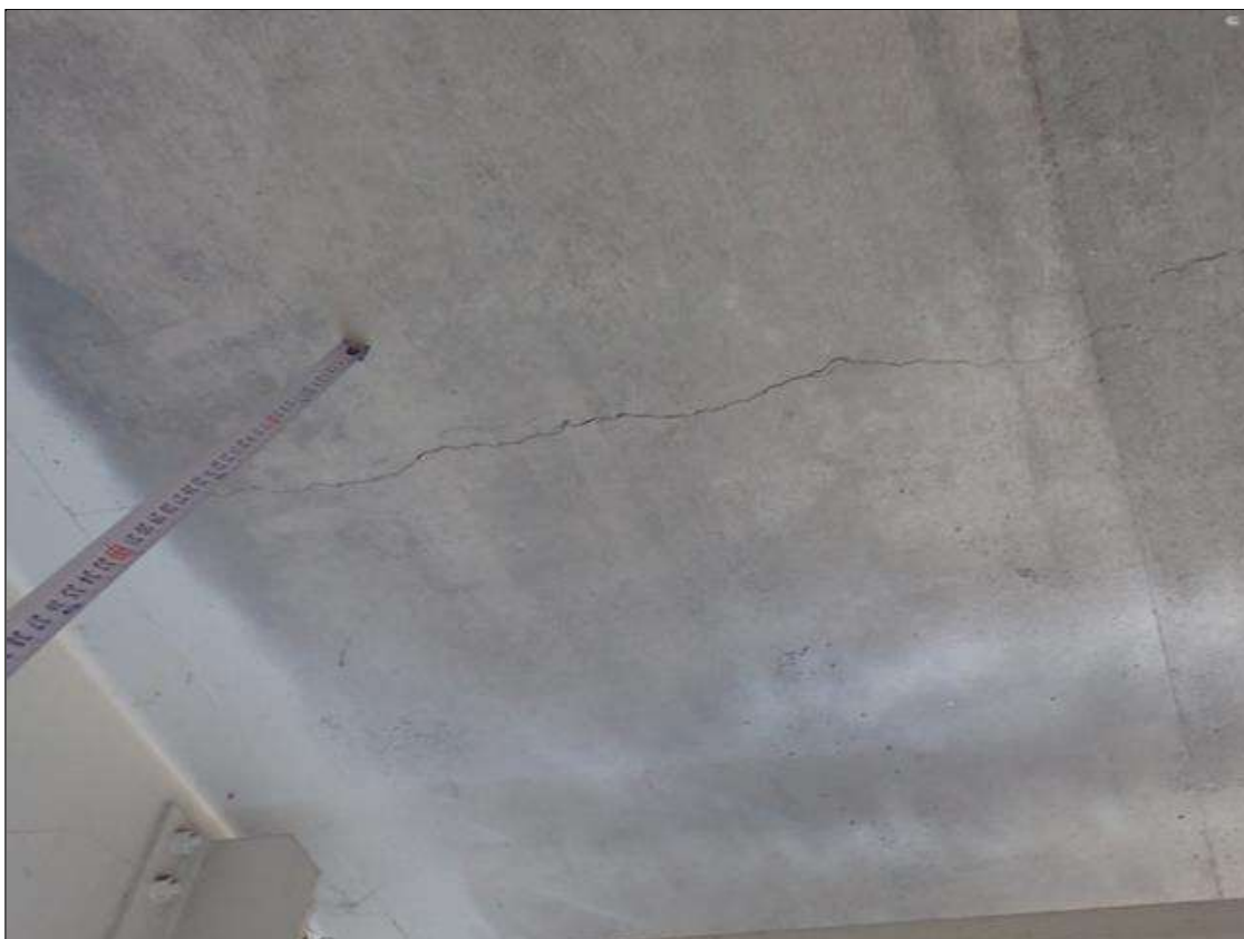
Span 1 Deck: throughout underside of deck, transverse cracks (up to 1/16 inch x full bay width) and map cracks (1/32 inch) at random
