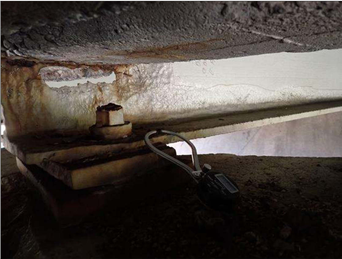
Span 4 Beam 5: (PAR) at bent 3, painted over section loss: web (1/4 inch average remaining x 6 foot x 1 foot) with corrosion holes (6 inch x 1.5 inch); bottom flange (0.56 inch average remaining x 15 inch) with corrosion reinitiated
