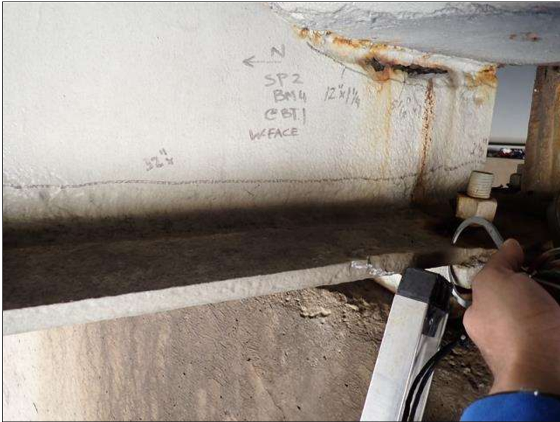
Span 2 Beam 4: (PAR) at bent 1, painted over section loss: web adjacent to diaphragm (1/4 inch average remaining x 12 inch x 2.5 inch) with corrosion hole (6 inch x 1 inch); lower web (5/16 inch average remaining x 52 inch x 2 inch); bottom flange (0.55 inch average remaining x 10 inch) with corrosion reinitiated
