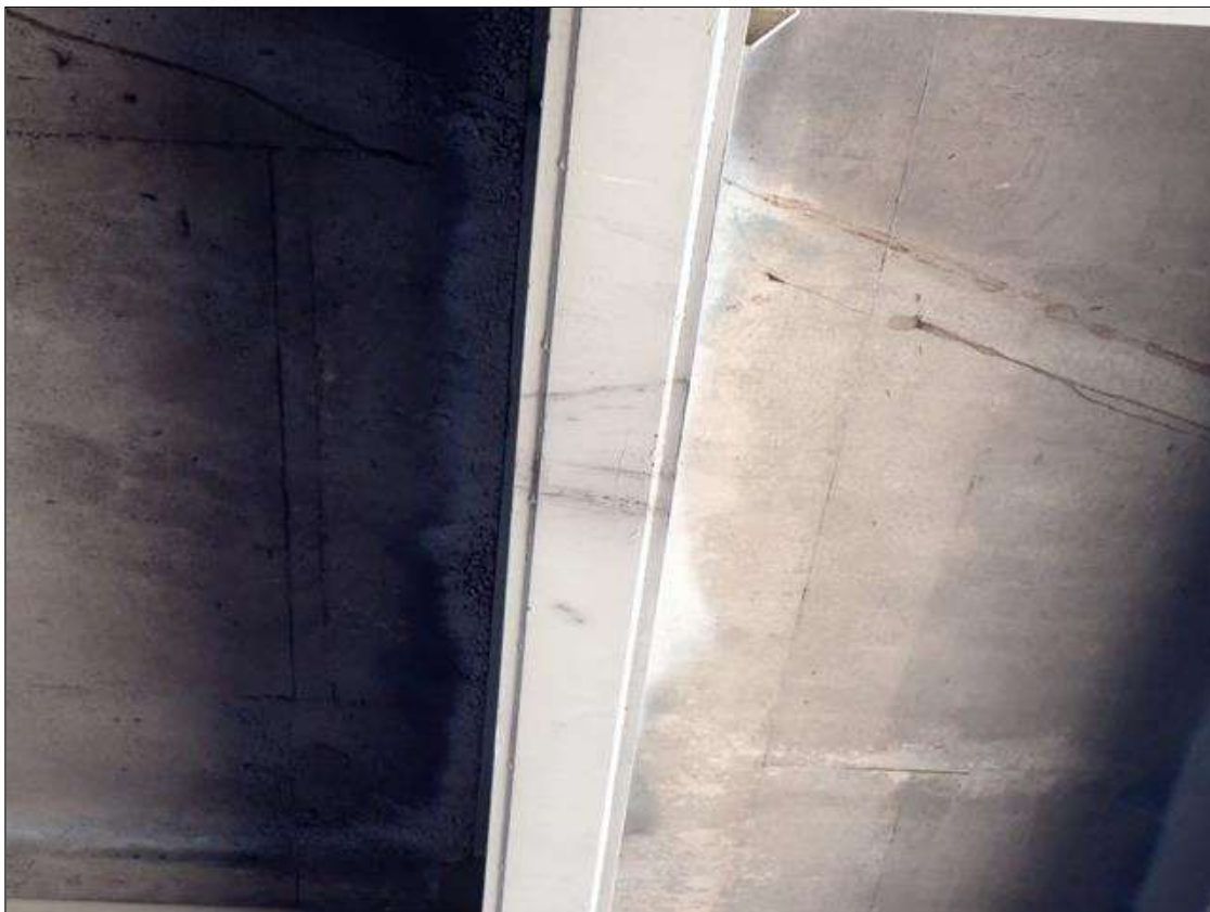
Span 3 Beam 4: (2023 no apparent change since previous inspection) SUPPLEMENTAL INSPECTION IMPACT DAMAGE 2021: scattered scrapes
