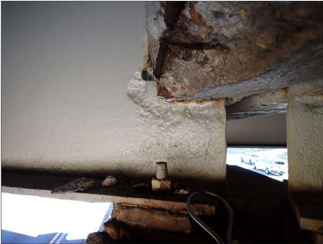
Span 3 Beam 5: (PAR) at bent 2, painted over section loss: bottom flange (0.60 inch average remaining x 3 foot); web (1/4 inch average remaining x 3 foot x 12 inch) with hole (1.5 inch x 1 inch) with corrosion reinitiated
