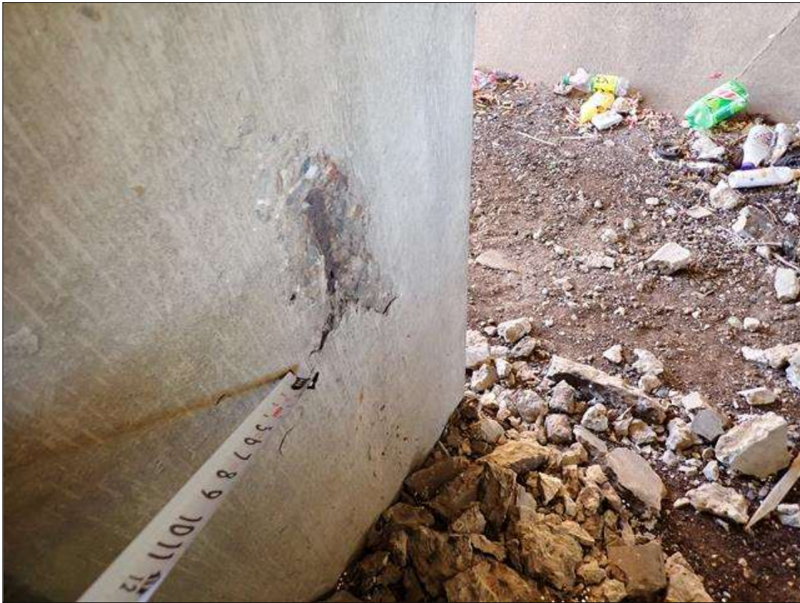
Bent 3 Pile 3: east face 12 inch high x 6 inch wide x 1 inch deep spall with exposed reinforcement
