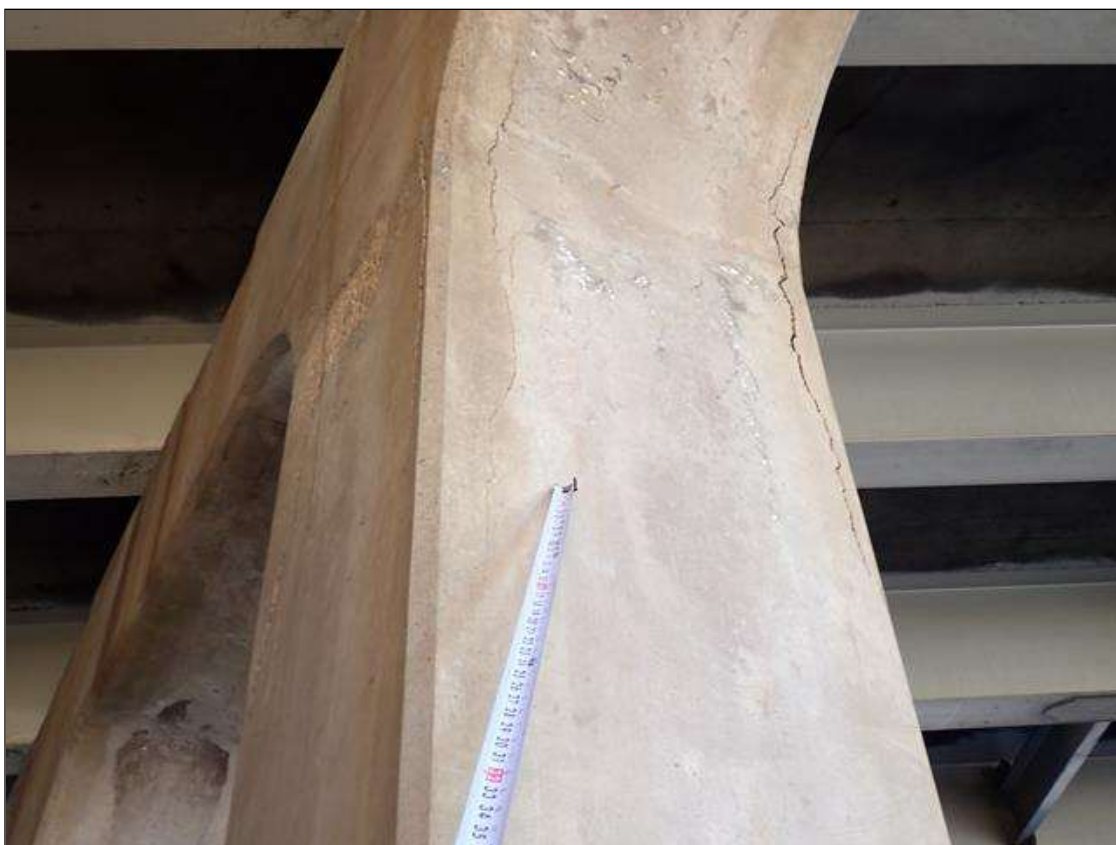
Bent 3 Pile 4: 29 inch wide x height varying from 18 inch to 45 inch area of delamination on west face. 3 foot high x 12 inch wide area of delamination in south face. 3 foot high x 12 inch wide area of delamination in north face.
