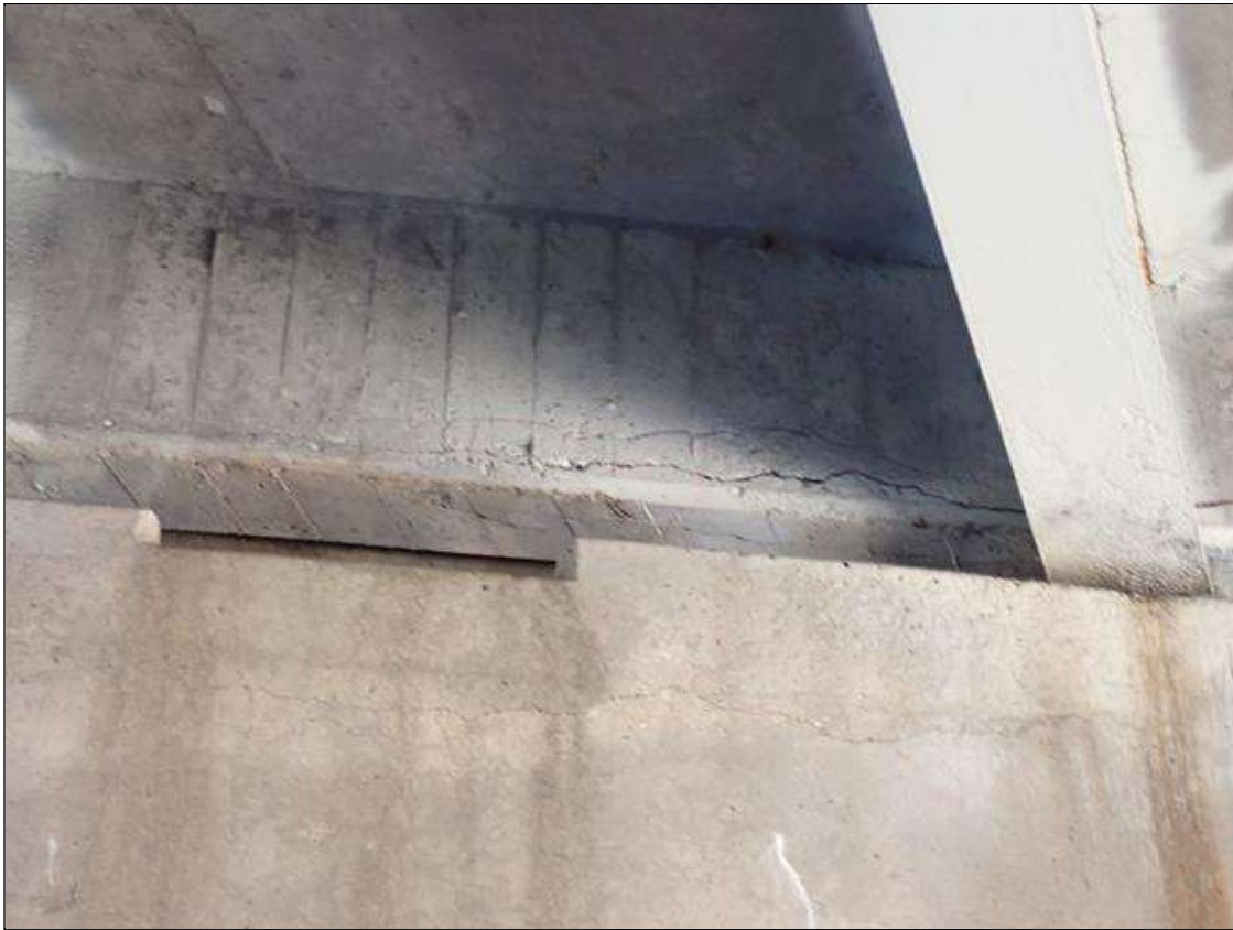
Span 4 Beam 5: 4 foot x 6 inch long x 8 inch wide x 5 inch along north and bottom faces area of delamination and unsound concrete in end diaphragm at bent 3 between beams 5 and 6.
