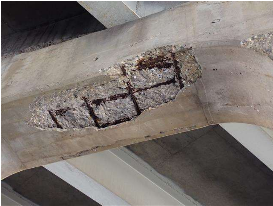
Bent 2 Cap 1: [PAR] bottom face of cap between columns 4 and 5, spall/delamination [5 foot long x full width x up to 3 inch deep] with seven exposed rusted reinforcing with 80 percent remaining
