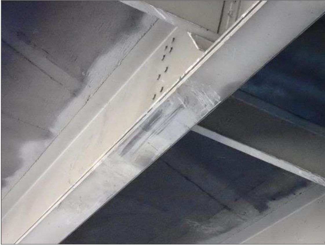
Span 3 Beam 9: (2023 no apparent change since previous inspection) SUPPLEMENTAL INSPECTION IMPACT DAMAGE 2021: 1 indentation 1 inch long x 1/4 inch deep at 18 foot-7 inch from interior. bent 3
