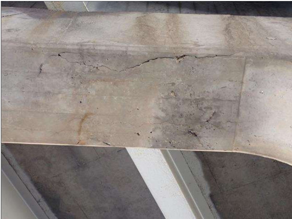
Bent 2 Cap 1: between columns 3 and 4, 4 foot long x full width delamination in the bottom face extending into vertical faces of concrete
