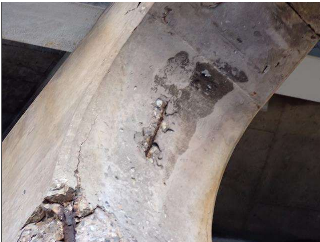
Bent 3 Cap 1: 12 inch x 4 inch x 1/2 inch deep spall with exposed reinforcement on east face of top radius at pile 5
