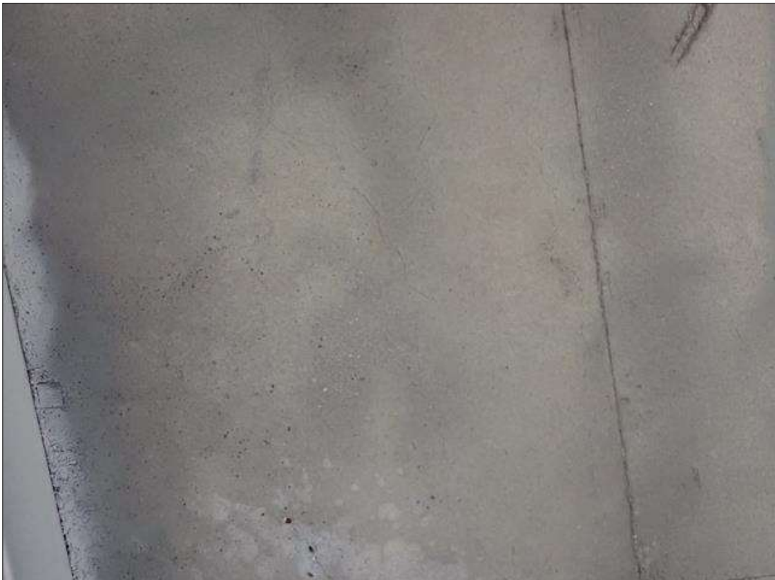
Span 2 Deck: throughout underside of deck, transverse cracks (up to 1/16 inch x full bay width) and map cracks (1/32 inch) at random
