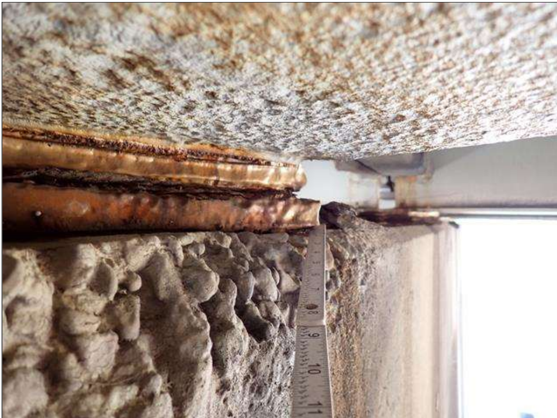
Span 3 Near Bearing 5: (PAR) loss of bearing area (up to 1/2 inch x 3 inch)
