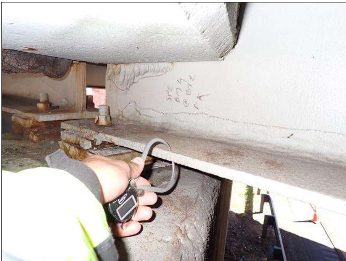
Span 2 Beam 4: (PAR) at bent 2, painted over section loss: bottom flange (0.60 inch average remaining x 2.5 foot), lower web (5/16 inch average remaining x 27 inch x 2 inch), web adjacent to diaphragm (1/4 inch average remaining x 11 inch x 3 inch) with corrosion reinitiated
