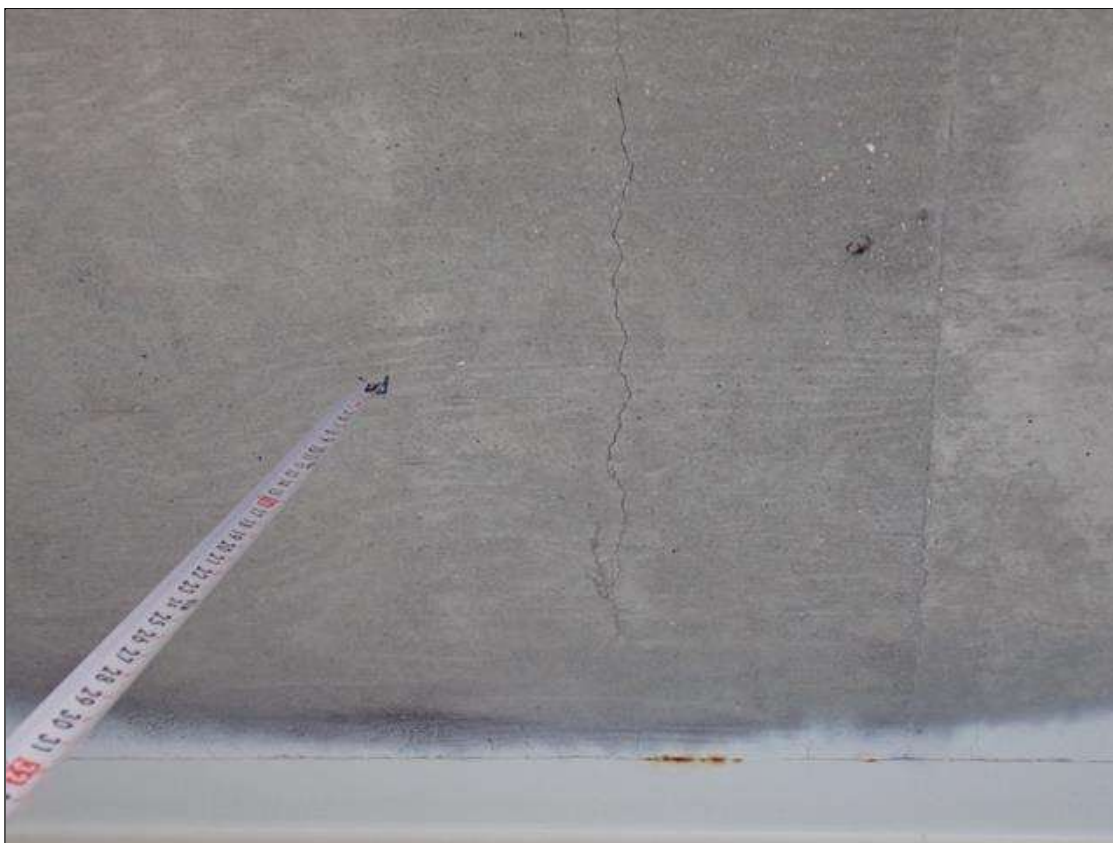
Span 1 Deck: throughout underside of deck, transverse cracks (up to 1/16 inch x full bay width) and map cracks (1/32 inch) at random
