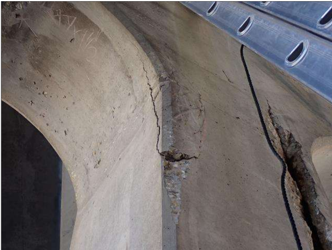
Bent 2 Pile 3: southwest corner, below cap, spall/delamination (36 inch x 10 inch x 1 inch deep)
