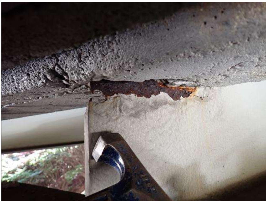
Span 1 Beam 7: (PAR) at bent 1 active corrosion with section loss, web at diaphragm [10 inch x 2 inch x 3/16 inch average remaining] with 1/2 inch diameter corrosion hole
