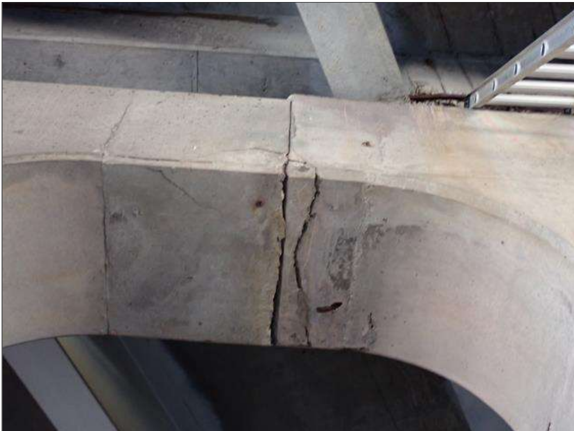
Bent 1 Cap 1: 1 foot long x full width of cap area of delaminated concrete with cracks up to 1/8 inch extends 1 foot into north face between columns 5 and 6.
