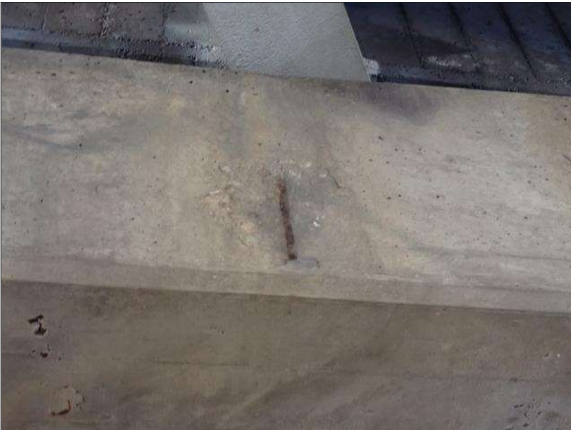
Bent 3 Cap 1: 12 inch high x 9 inch wide x 1.5 inch deep with exposed reinforcement under beam 7, south face. 90 percent section remaining in exposed reinforcement.
