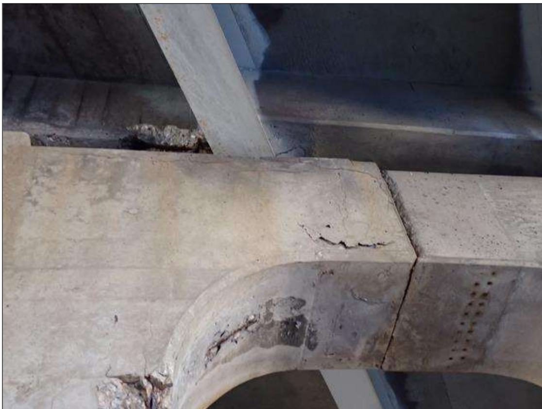
Bent 3 Cap 1: 5 foot x up to full height area of cracked delamination on south face of cap below beam 8
