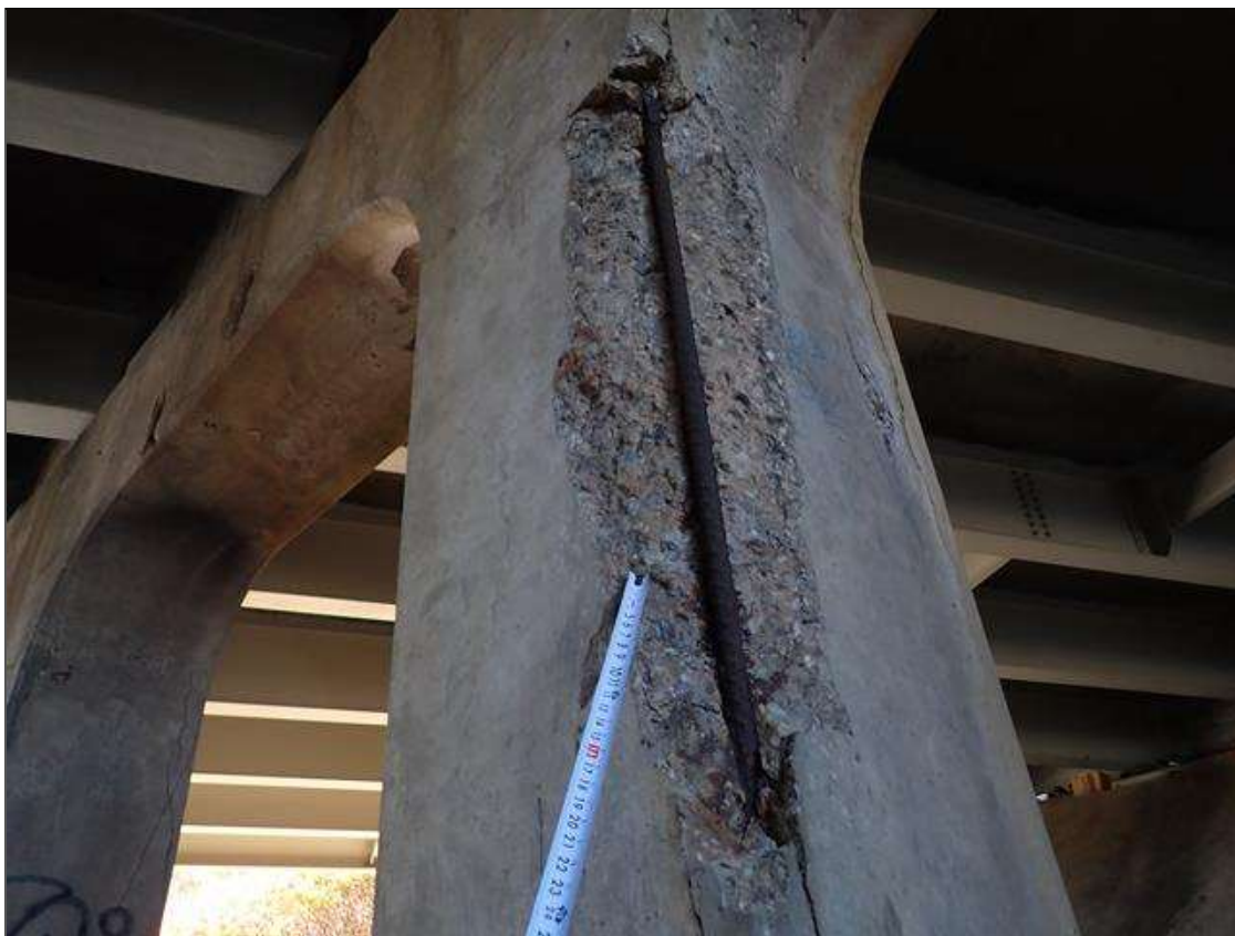
Bent 3 Pile 5: (PAR) 6.5 foot high x 20 inch wide x 3.5 inch deep spall and delaminated concrete with one debonded primary exposed reinforcement on south east corner of pile. 80 percent section remaining in exposed reinforcement.
