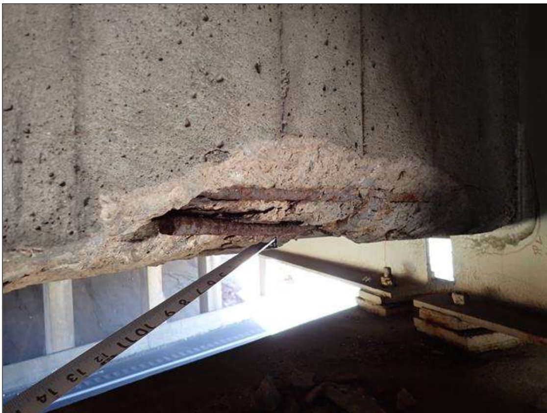
Span 2 Beam 7: (PAR) 2 foot x 4 inch x 3 inch deep spall with exposed rusted and debonded reinforcement on south face of end diaphragm, at bent 2
