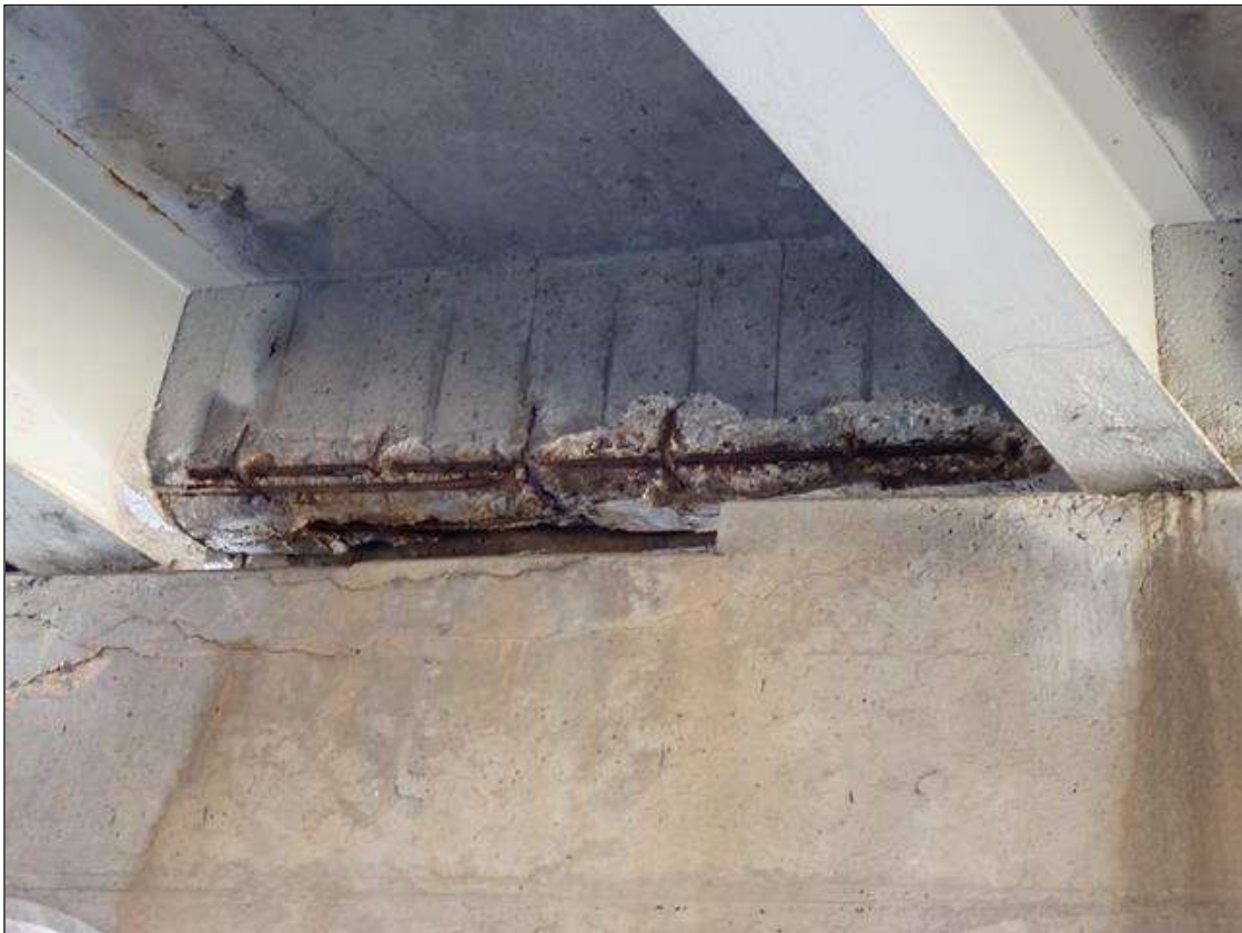
Span 4 Beam 8: (PAR) 7 foot long x 1.5 foot wide x 3 inch deep spall with exposed reinforcement in end diaphragm between beams 7 and 8 at bent 3. 60 percent section remaining in exposed reinforcement.
