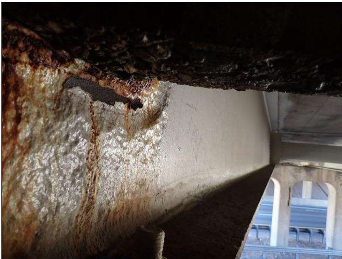
Span 2 Beam 4: (PAR) at bent 1, painted over section loss: web adjacent to diaphragm (1/4 inch average remaining x 12 inch x 2.5 inch) with corrosion hole (6 inch x 1 inch); lower web (5/16 inch average remaining x 52 inch x 2 inch); bottom flange (0.55 inch average remaining x 10 inch) with corrosion reinitiated
