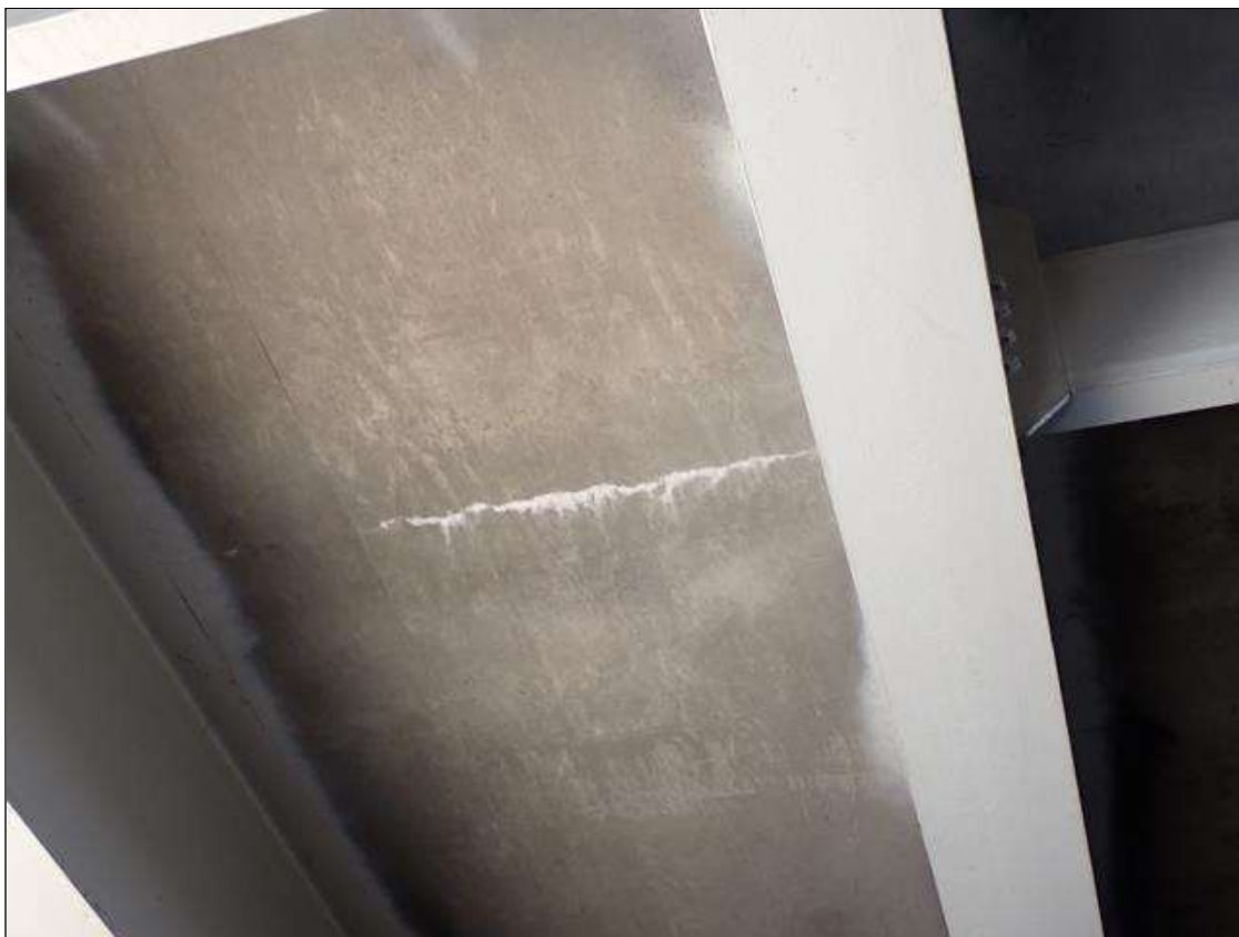
Span 4 Deck: throughout underside of deck, transverse cracks (up to 1/16 inch x full bay width) and map cracks (1/32 inch) some with efflorescence at random
