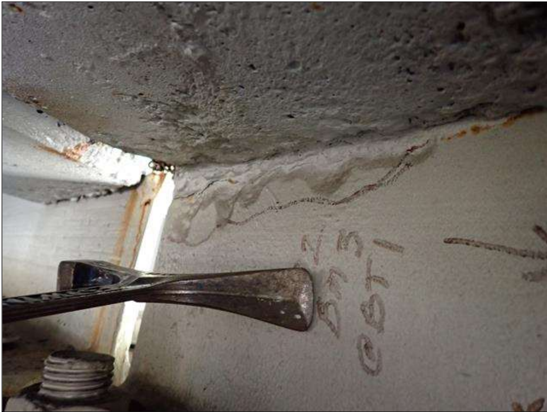
Span 2 Beam 3: (PAR) 10 inch long x up to 2 inch high x 5/16 inch section remaining in the web at beam end at bent 1, spot rust present
