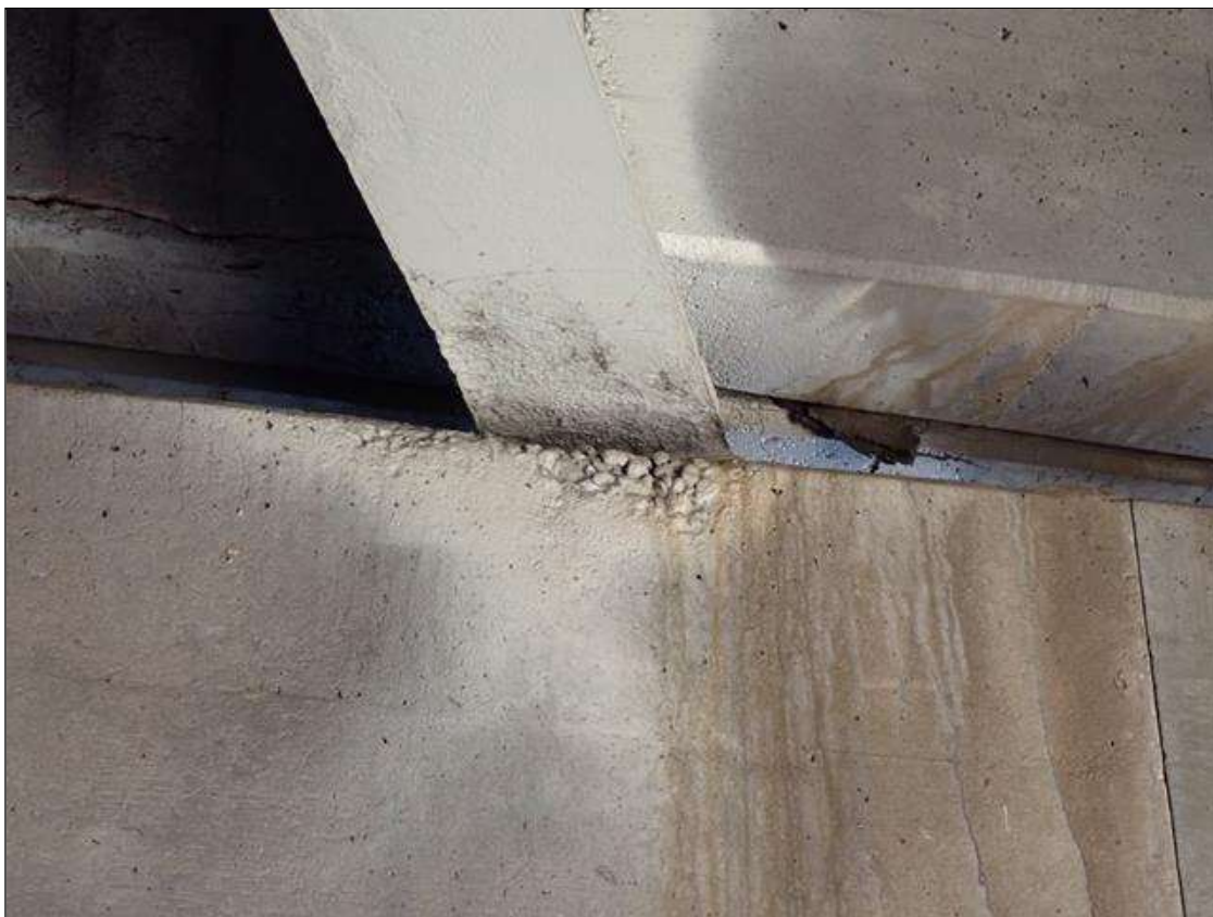
Bent 3 Cap 1: North face under beam 4, spall [1 foot x 6 inch x 1/2 inch deep] no undermining
