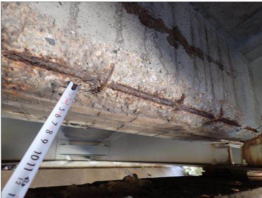
Span 2 Beam 5: (PAR) 7 foot long x 10 inch high x 3 inch wide area of spall, delamination with exposed reinforcement in the concrete diaphragm between beams 5 and 6 at bent 1. 70 percent section remaining in the exposed reinforcement
