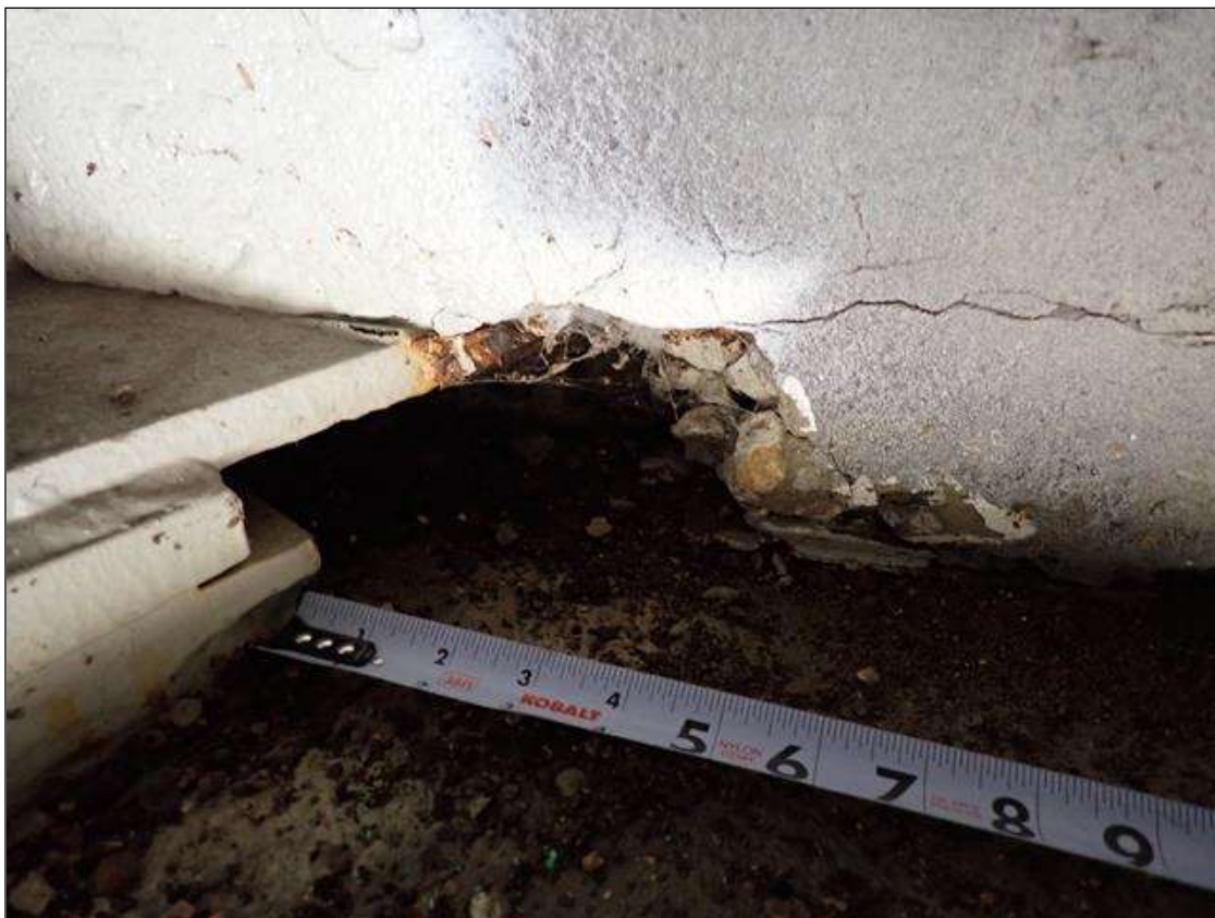
End Bent 1 Abutment: along the length of the abutment, adjacent to beam bottom flanges, spall/delaminations (up to 9 inch x 4 inch x 4 inch deep) with cracks (up to 1/8 inch)
