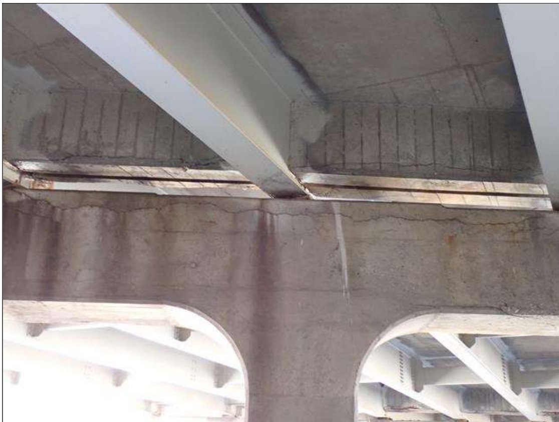
Bent 1 Cap 1: 15 foot long x 12 inch delamination with cracks up to 1/8 inch between beams 5 and 7 on south face of the cap.
