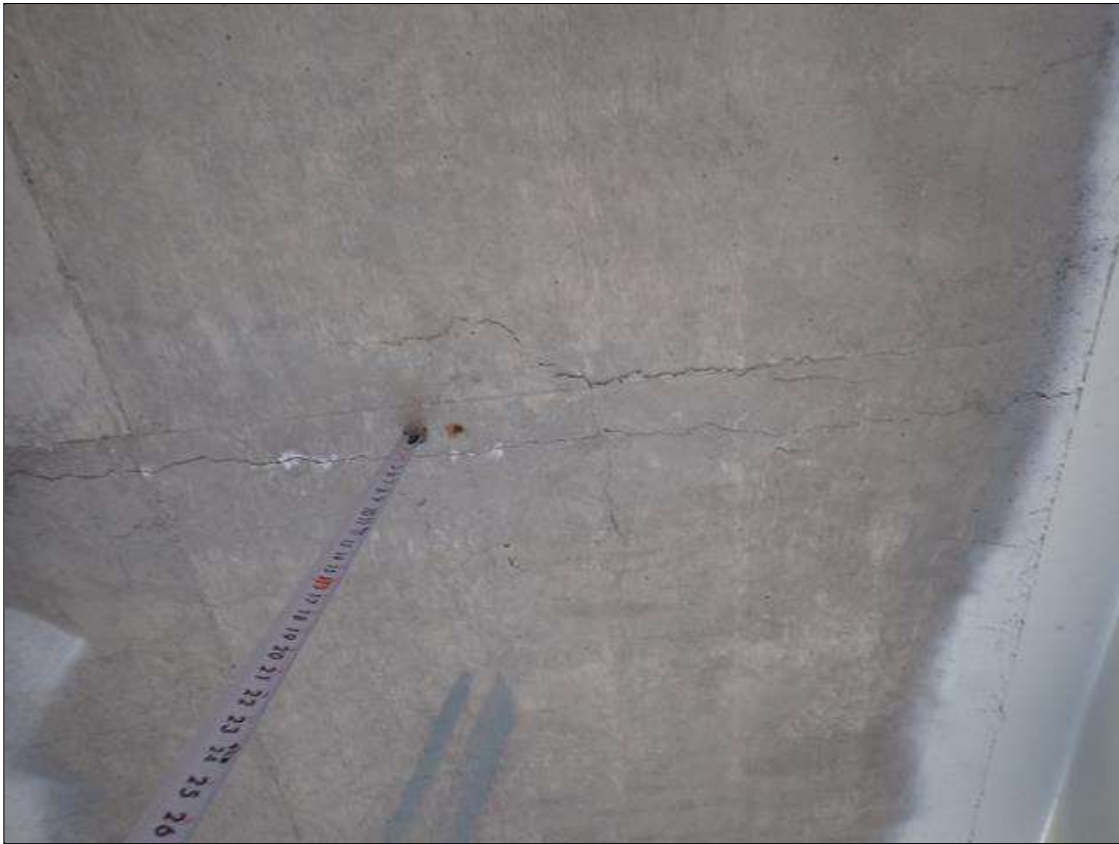
Span 1 Deck: underside of deck, bay 2, at end bent 1 and midspan, (2) delaminations (up to 3 foot x 1 foot)
