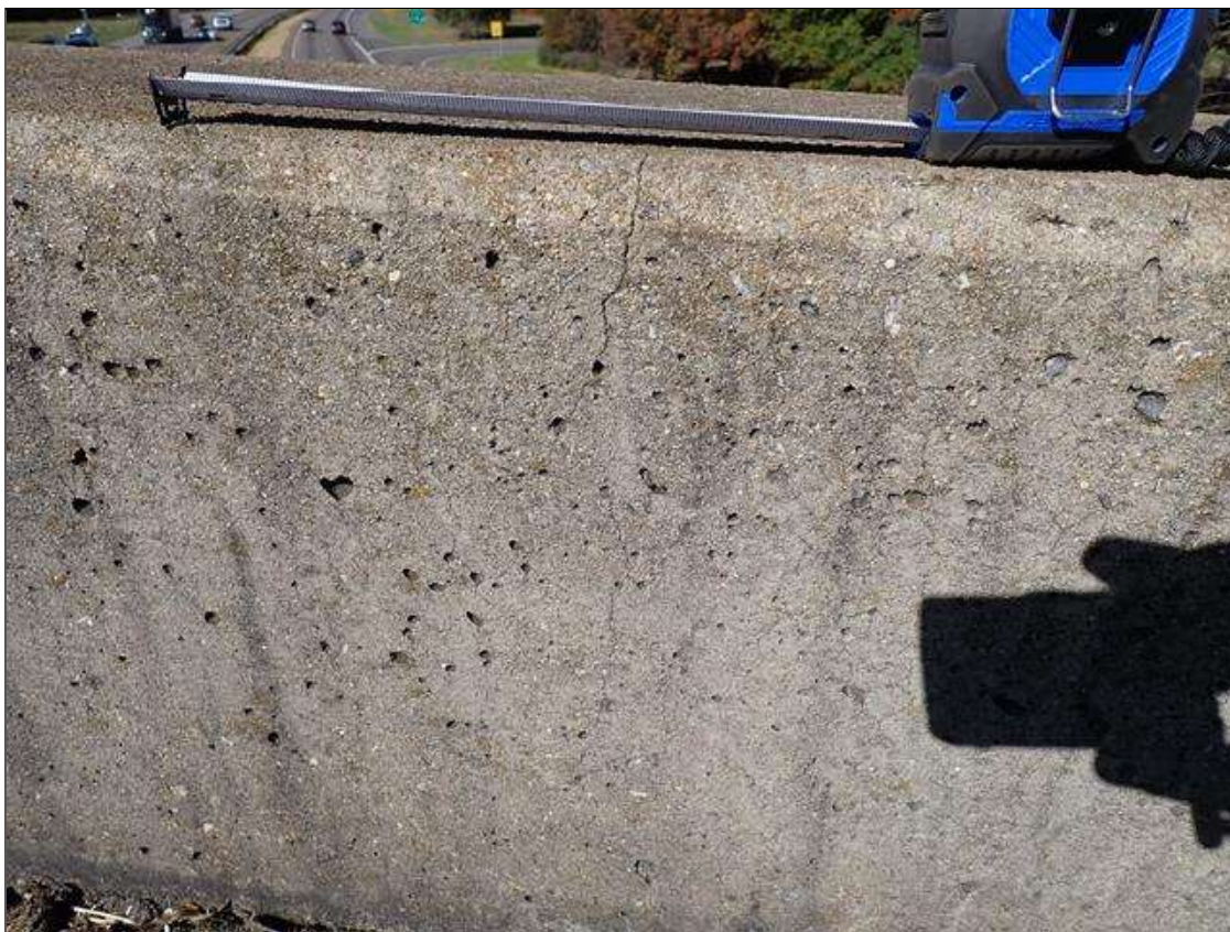
Span 3 Left Bridge Rail: along the length of parapet, vertical cracks (up to 1/32 x full height) at random
