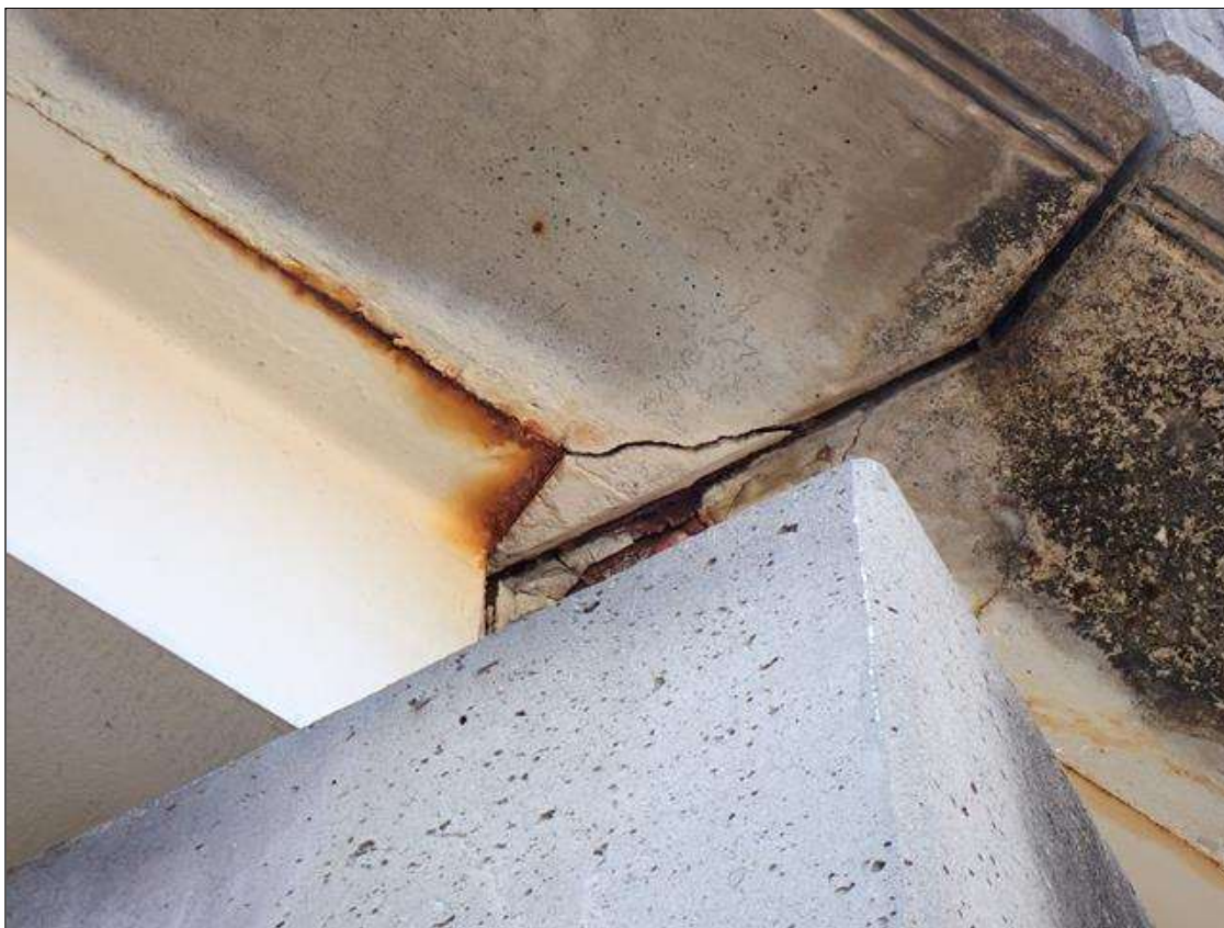
Span 3 Deck: at bent 3, both overhangs, (2) delaminations (up to 1.5 foot x 6 inch)
