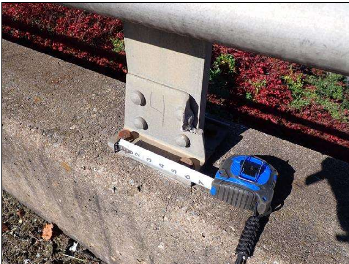
Span 1 Left Bridge Rail: (PAR) impact damage to rail bracket of fourth post
