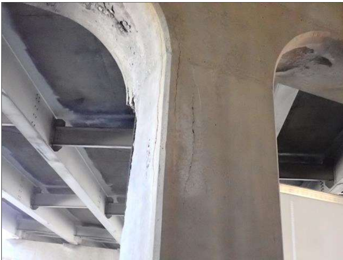
Bent 3 Pile 5: 4 foot high x 16 inch wide area of delamination/spall and unsound concrete at northeast corner.
