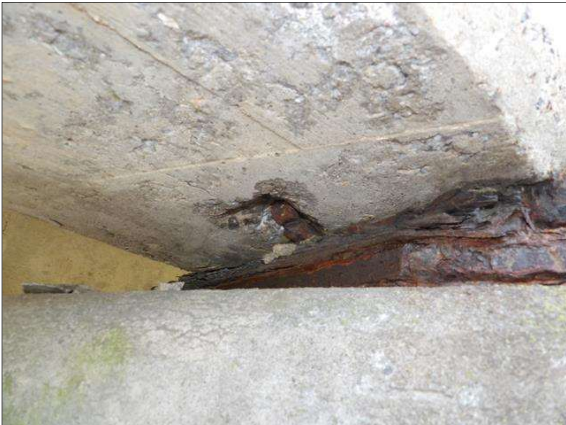
Span 2 Beam 5: 4 INCHES LONG X 4 INCHES WIDE X 1 INCHES DEEP SPALL ON BOTTOM FACE OF BEAM WITH EXPOSED STEEL NO LOSS AT FAR BEARING
