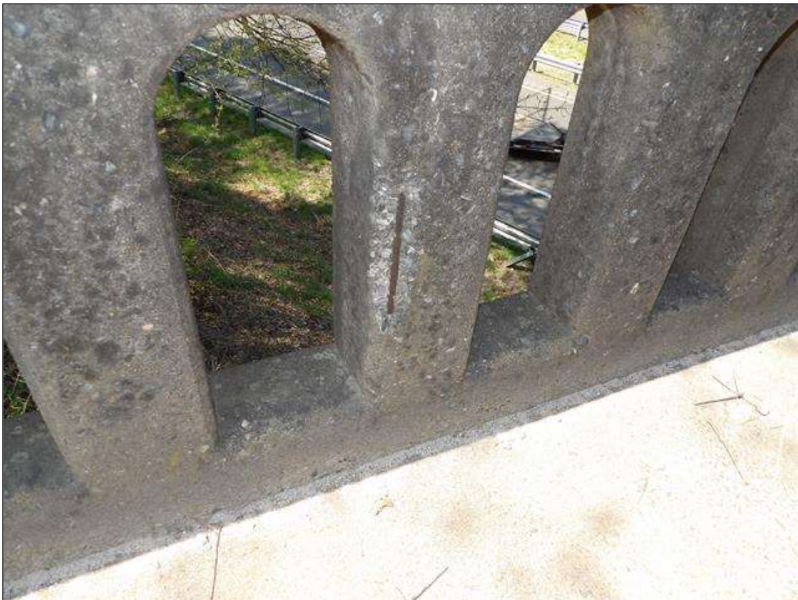
TYPICAL-- SPALLS UP TO 19 INCHES HIGH X 2 INCHES WIDE X 0.5 INCHES DEEP WITH EXPOSED REBAR THROUGHOUT FRONT AND BACK FACE OF BARRIER RAIL PEDESTALS SPAN 1 LEFT SHOWN
