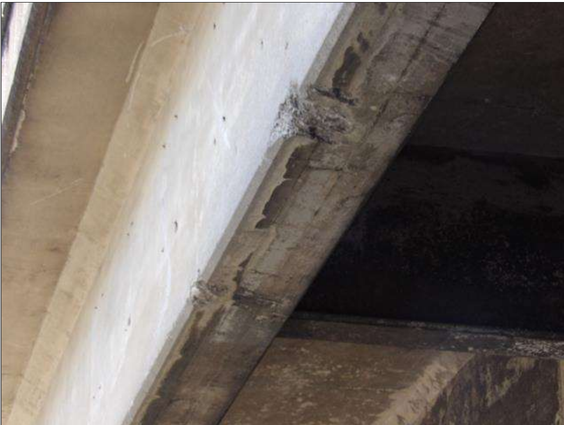
Span 2 Beam 1: (2) HIGH HIT SPALLS UP TO 18 INCHES LONG X 9 INCHES (BOTTOM FACE) X 4 INCHES (WEB) X 1 INCHES DEEP AT BOTTOM LEFT CORNER OF BEAM 1 NEAR MIDSPAN
