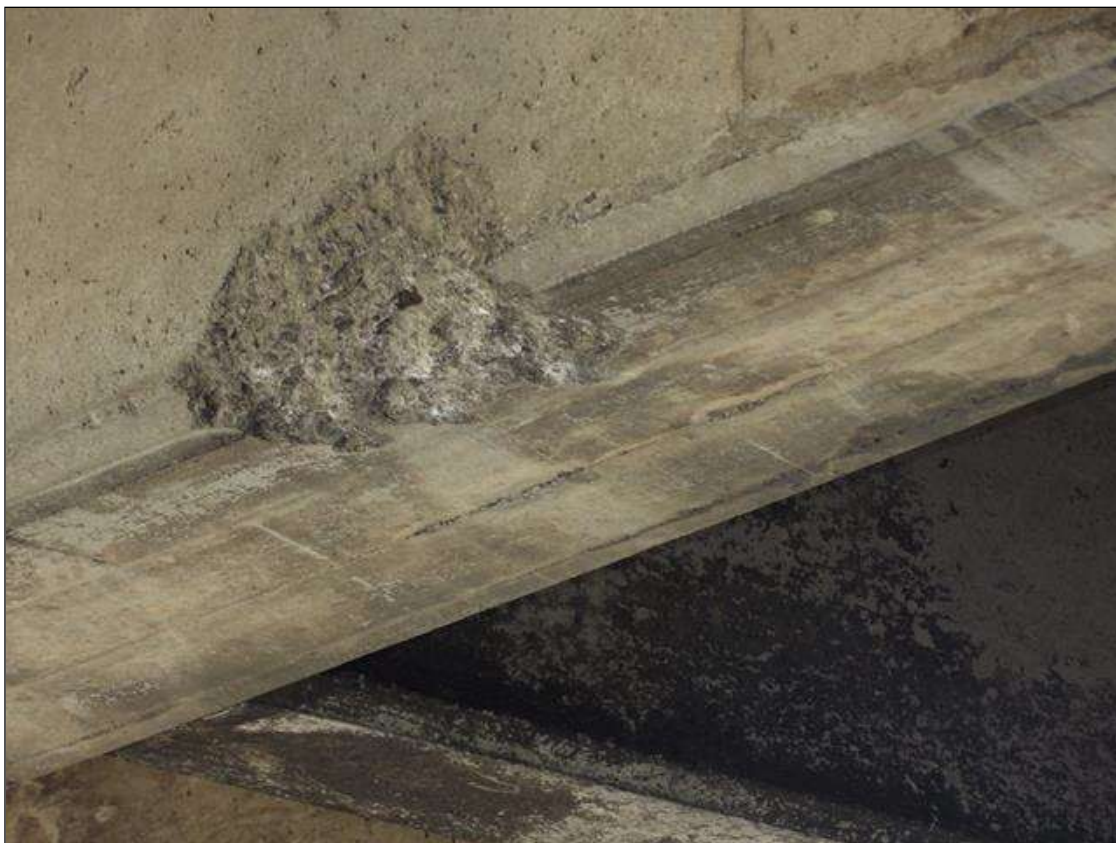
Span 2 Beam 2: IMPACT SPALL 15 INCHES LONG X 6 INCHES (BOTTOM FACE) X 6 INCHES (WEB) X 3 INCHES DEEP AT BOTTOM CORNER OF BEAM 2 NEAR MIDSPAN
