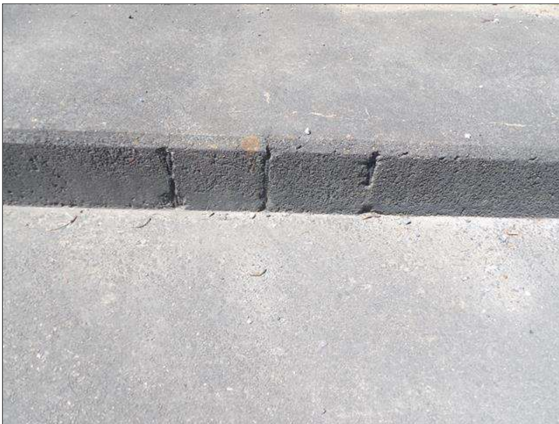
SPAN 2 LEFT SIDEWALK (3) 9 INCHES HIGH X 3/4 INCHES WIDE X 1/4 INCHES DEEP SPALLS WITH EXPOSED REBAR ON VERTICAL FACE OF LEFT SIDEWALK , APPROXIMATELY 15 FEET FROM BENT 1
