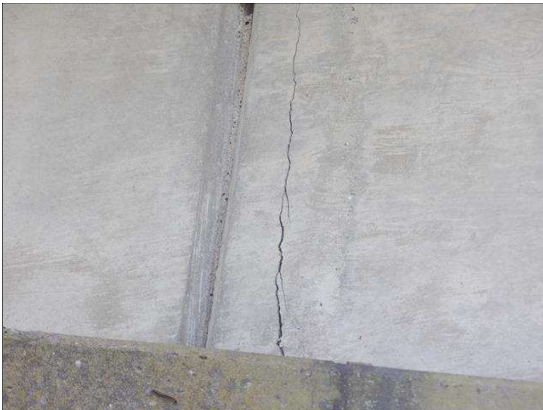
Span 2 Beam 5: AT BENT 1, 30 INCHES HIGH VERTICAL CRACK UP TO 1/8 INCHES WIDE EAST FACE
