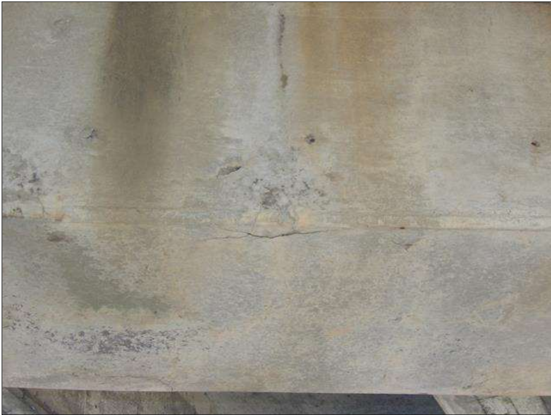
Bent 3 Cap 1: 16 INCHES LONG X 6 FEET HIGH AREA OF DELAMINATION WITH CRACKING UP TO 0.0625 INCHES WIDE ON BOTTOM OF CAP AND EXTENDING UP FAR FACE UNDER BEAM 4
