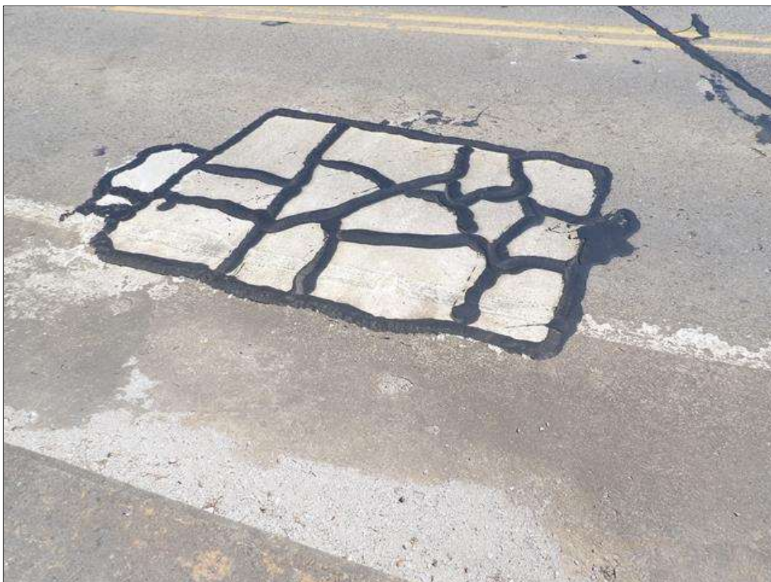
Span 3 Deck: 4.5 FEET WIDE X 7 FEET LONG SOUND PATCH WITH INTERMITTENT SEALED CRACKING IN SOUTHBOUND TRAVEL LANE NEAR BENT 2
