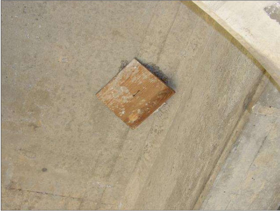
SPAN 4 DECK UNDERSIDE-- DECK REPAIR FORM LEFT IN PLACE (BAY 2, 6 FEET FROM BENT 3)
