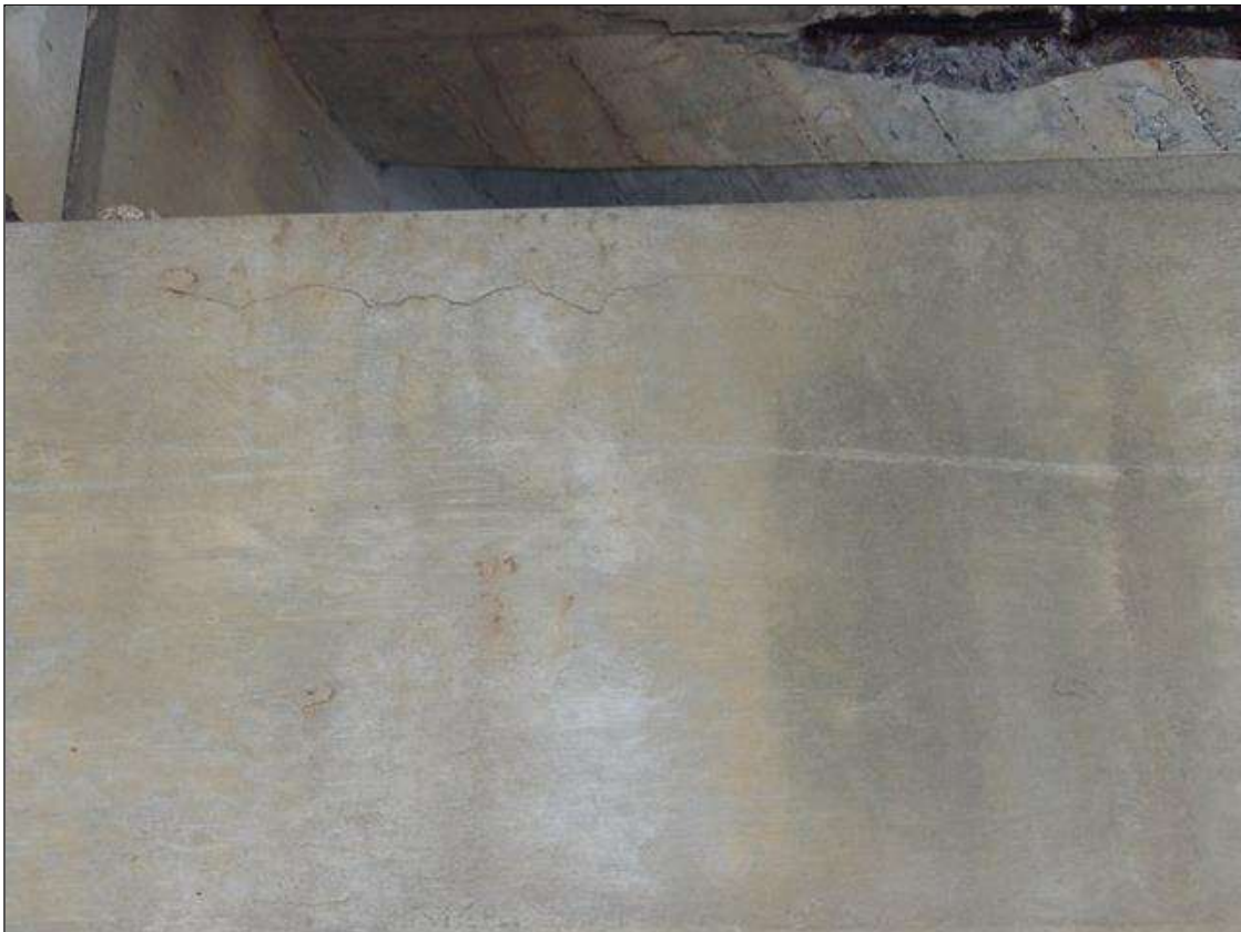
Bent 2 Cap 1: 2 FEET LONG HORIZONTAL CRACK 1/16 INCHES WIDE ON NEAR FACE IN BAY 2
