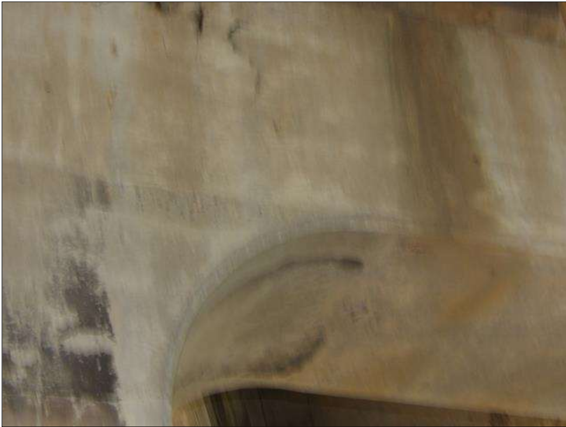
Bent 3 Cap 1: 3 FEET-6 INCHES LONG X 9 INCHES HIGH DELAMINATION, 6 INCHES DIAMETER X 1 INCHES DEEP SPALL WITH EXPOSED REBAR WITH ACTIVE CORROSION NO LOSS AND 5 INCHES HIGH X 1 INCHES WIDE X 3/4 INCHES DEEP SPALL WITH EXPOSED REBAR WITH ACTIVE CORROSION NO LOSS ON NEAR FACE UNDER BEAM 3
