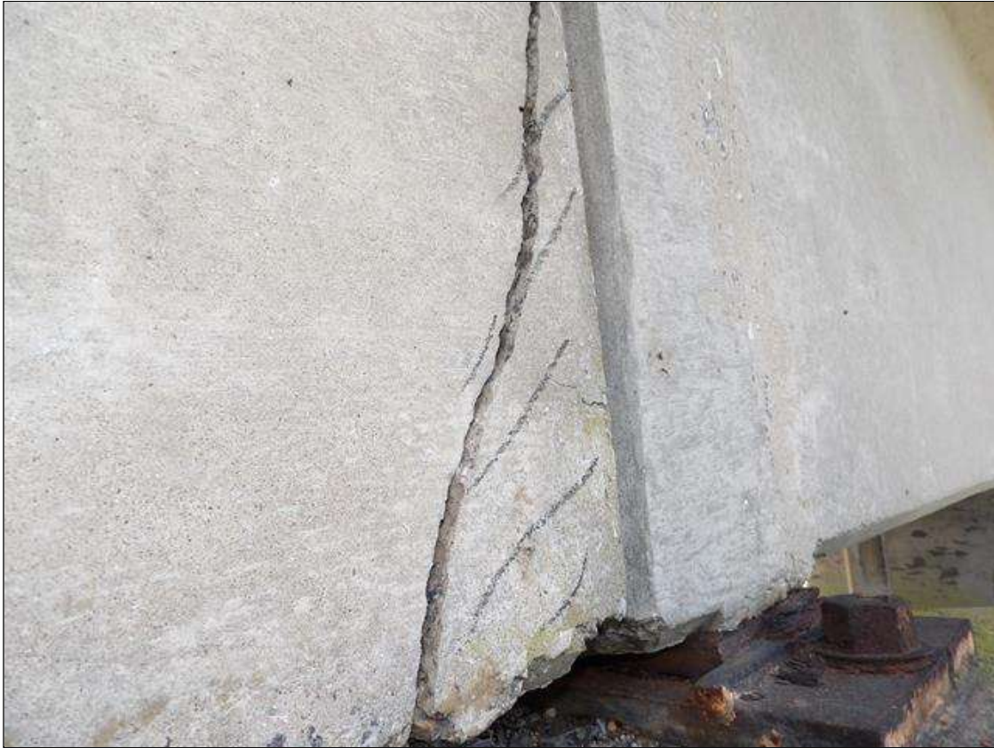
Span 2 Beam 5: AT BENT 2 BEARING, 24 INCHES HIGH X 6 INCHES WIDE DELAMINATION ON RIGHT SIDE, 1 FEET HIGH X 4 INCHES LONG ON LEFT SIDE, EXTENDING 3 INCHES ACROSS THE BEARING NO LOSS
