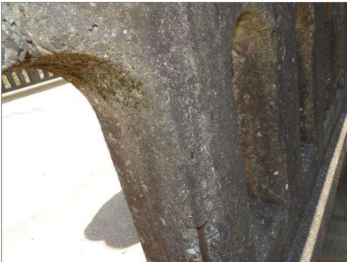
Span 2 Left Bridge Rail: PAR: (13) SPALLS AND DELAMINATED AREAS UP TO 2 FEET HIGH X 3 INCHES WIDE X 3 INCHES DEEP WITH EXPOSED REBAR INTERMITTENT THROUGHOUT FRONT AND BACK FACE OF BARRIER RAIL PEDESTALS, SOME AREAS ON BACK FACE ARE LOOSE AND OVER TRAFFIC
