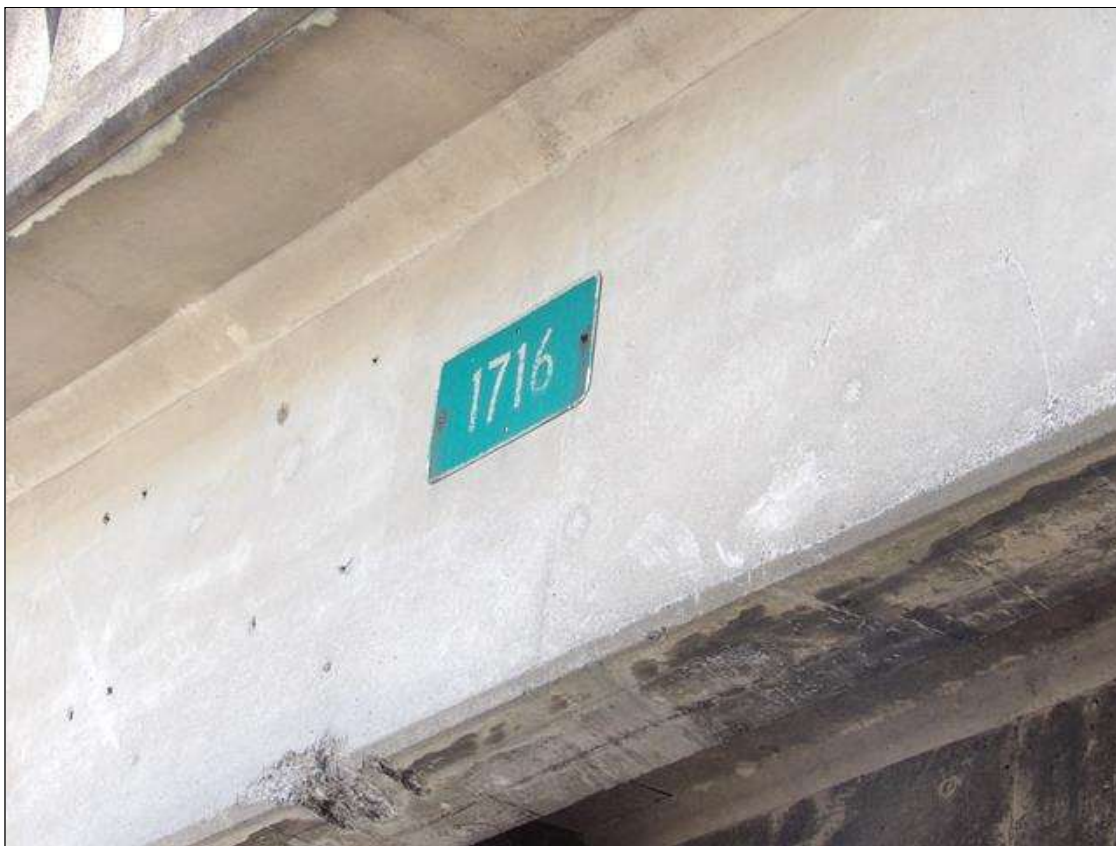
ROUTE 1716 SIGN REATTACHED TO SPAN 2 BEAM 1 WEST FACE TO FIX PREVIOUS PAR
