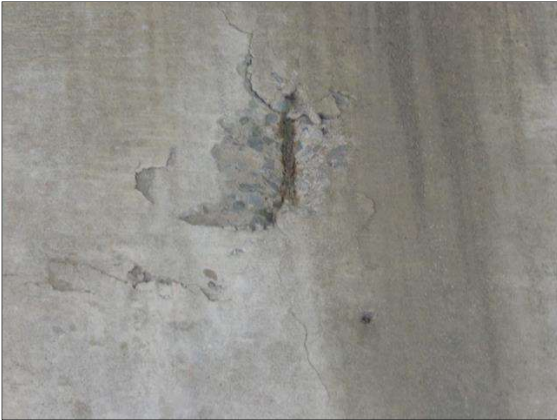
Bent 2 Cap 1: 2 FOOT-6 INCHES HIGH X 1 FOOT-6 INCHES WIDE X 1 1/4 INCHES DEEP SPALL WITH EXPOSED REBAR/AREA OF DELAMINATION WITH ACTIVE CORROSION NO LOSS ON NEAR FACE UNDER BEAM 3
