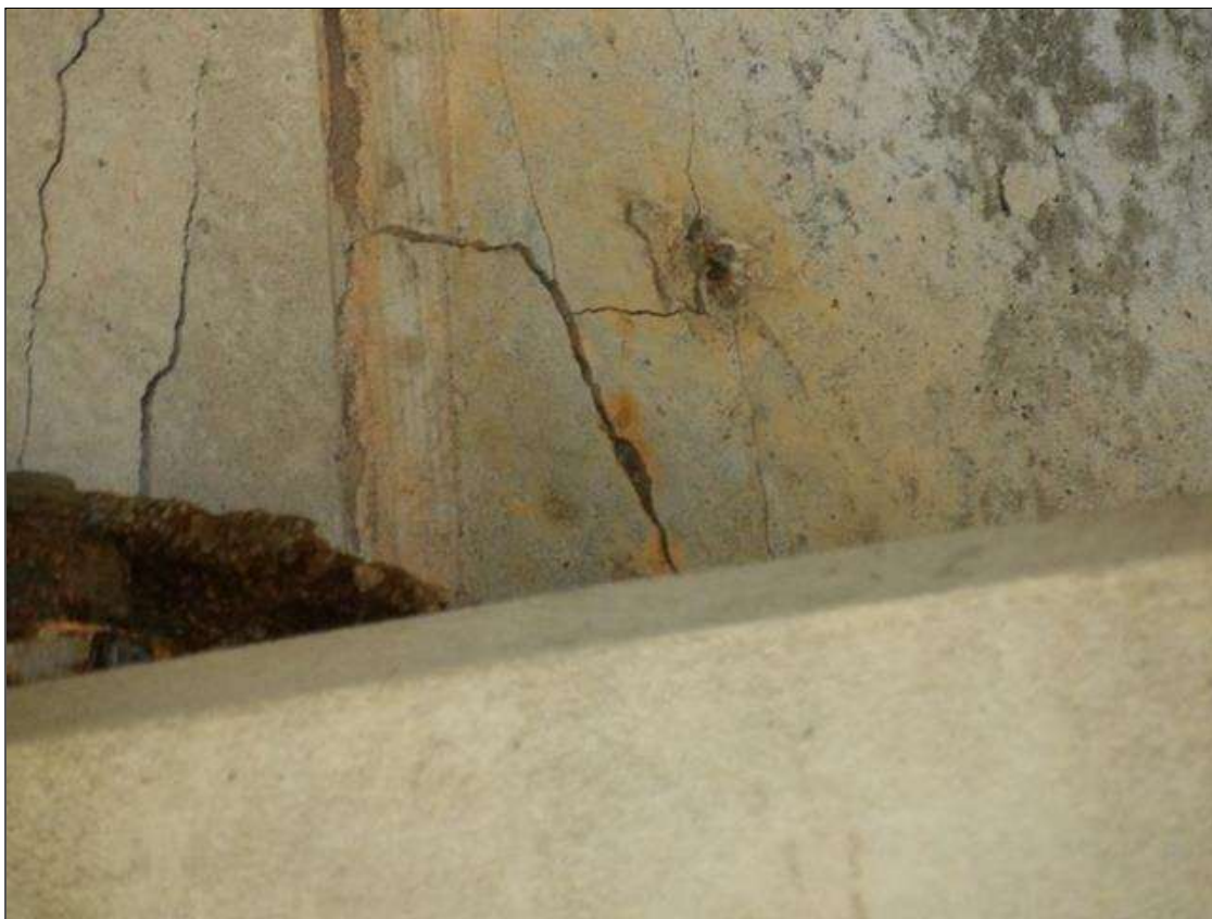
Span 3 Beam 4: AT BENT 3, 2 FEET HIGH X 6 INCHES WIDE DELAMINATED AREA ON LEFT SIDE
