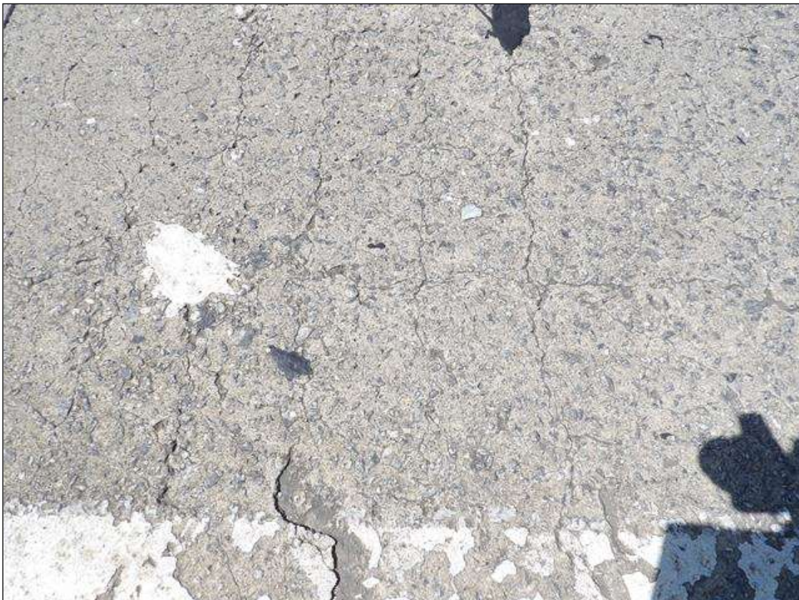
Span 4 Deck: UP TO 1/8 INCH WIDE TRANSVERSE CRACKS AT VARIOUS LOCATIONS IN TOP OF DECK
