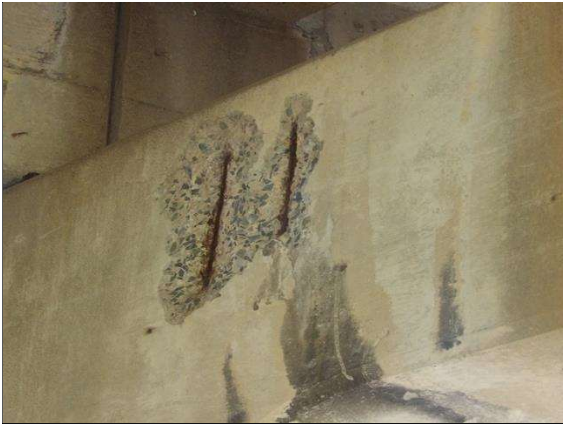
Bent 1 Cap 1: 20 INCHES HIGH X 20 INCHES WIDE X 1.5 INCHES DEEP SPALL WITH EXPOSED REBAR WITH ACTIVE CORROSION NO LOSS ON NEAR FACE IN BAY 1
