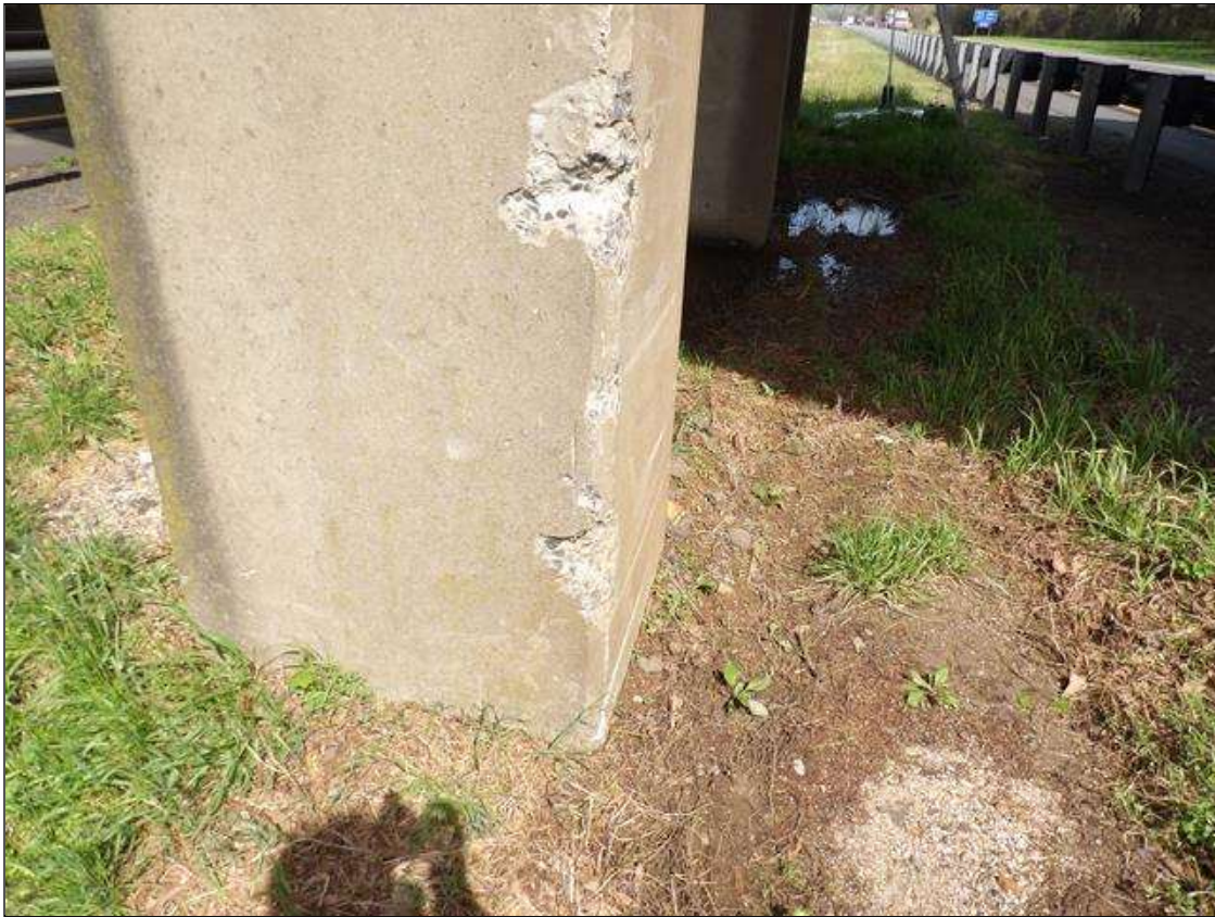
Bent 2 Pile 1: 3 SPALLS UP TO 12 INCHES X 4 INCHES X 4 INCHES AT NEAR LEFT CORNER NEAR BASE OF COLUMN 1
