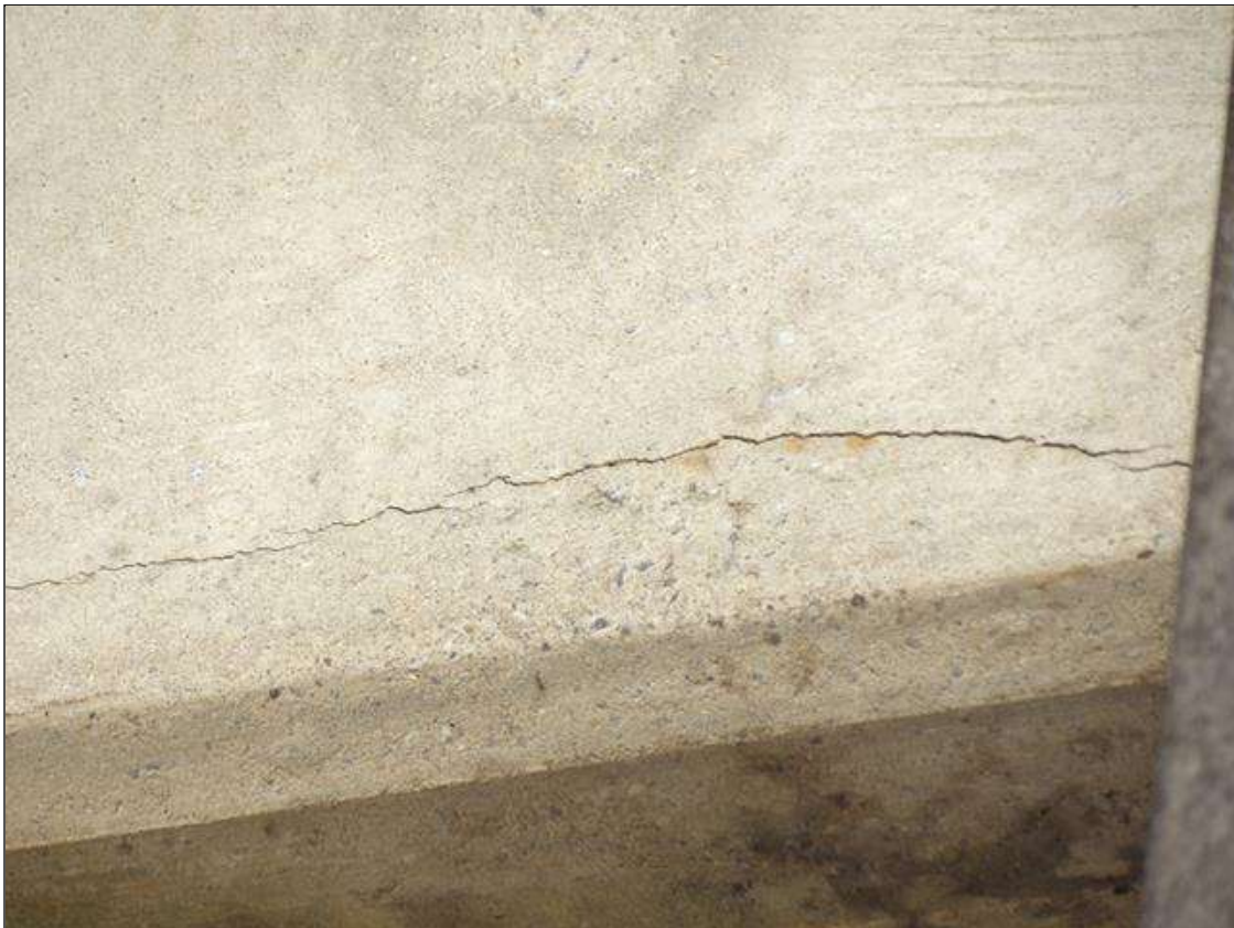
Span 2 Beam 1: AT BENT 1, UP TO 1/16 INCHES WIDE HORIZONTAL CRACK UP TO 3 FEET LONG IN LEFT FACE AT BOTTOM OF BEAM
