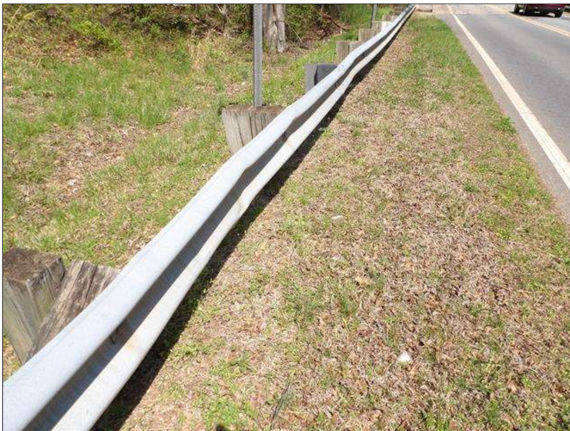
SOUTHWEST GUARDRAIL IMPACT DAMAGE 15 FEET LONG 20 FEET FROM TERMINAL END
