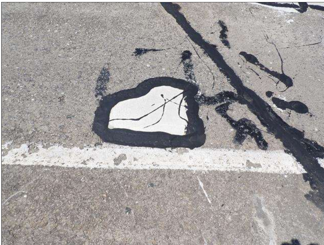
Span 3 Deck: SOUND PATCH TO FIX PREVIOUS PAR 18 INCHES LONG X 14 INCHES WIDE IN NORTHBOUND LANE 2 FEET FROM BENT 3 JOINT
