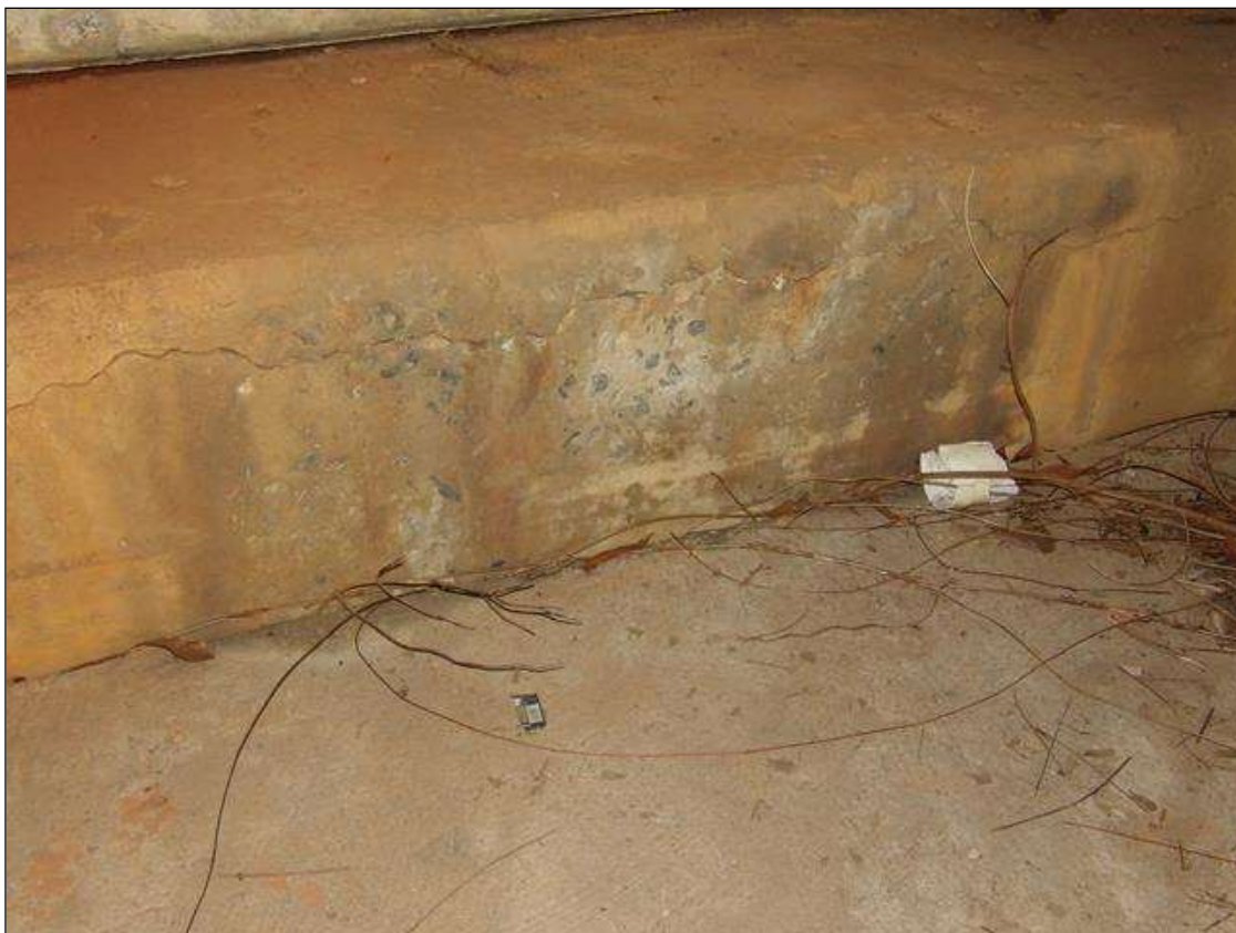
End Bent 2 Cap 1: 78 INCHES LONG HORIZONTAL CRACK UP TO 1/8 INCHES WIDE ON BAY 3 FACE OF CAP
