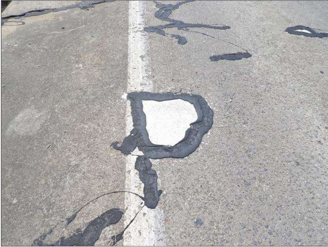
Span 3 Deck: SOUND PATCH TO FIX PREVIOUS PAR 18 INCHES DIAMETER LOCATED 6 FEET FROM BENT 2 IN THE NORTHBOUND TRAVEL LANE
