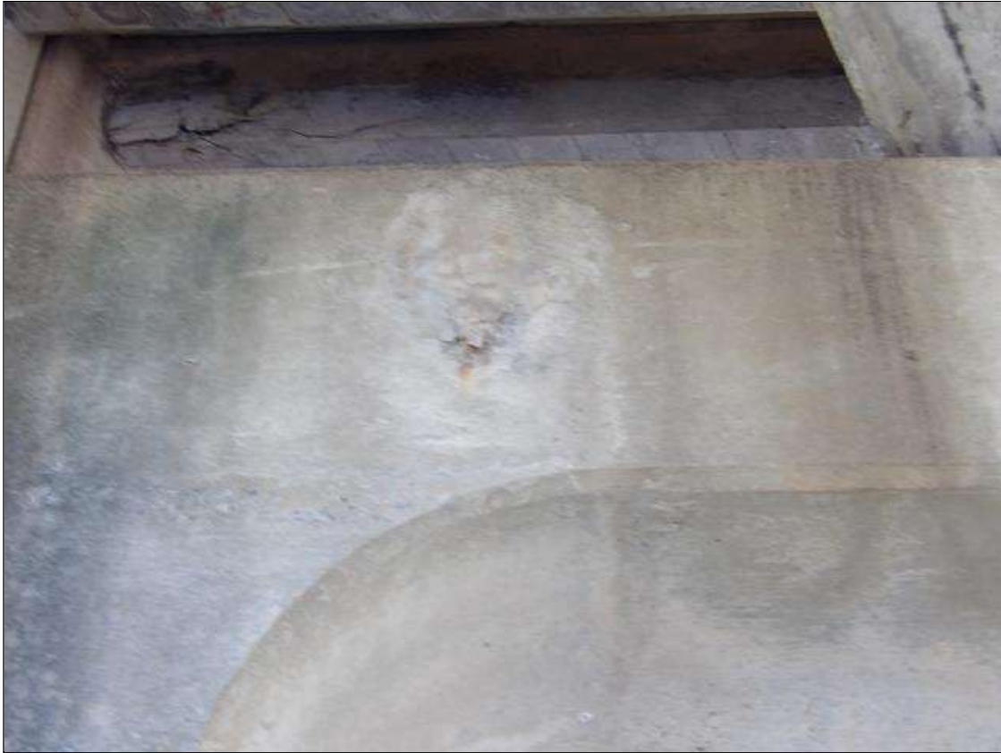
Bent 2 Cap 1: FAILED PATCHED AREA THAT IS 2 FEET DIAMETER X UP TO 3/4 INCHES DEEP ON FAR FACE UNDER BAY 4
