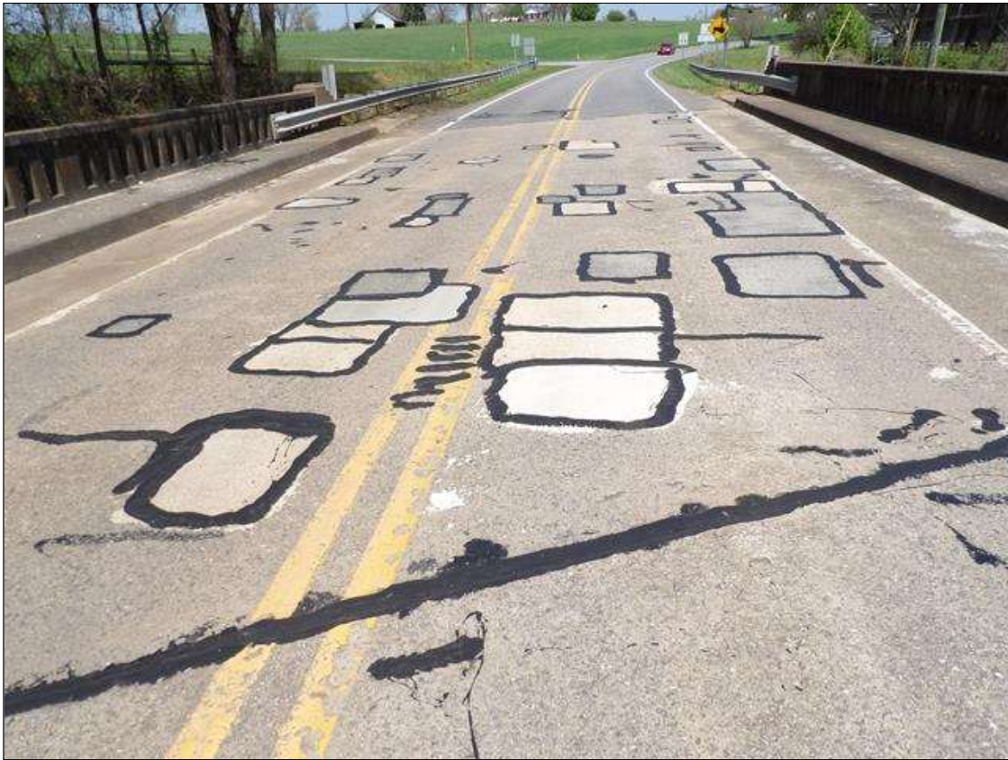
TYPICAL SOUND PATCHED AREAS IN SPAN 4 DECK
