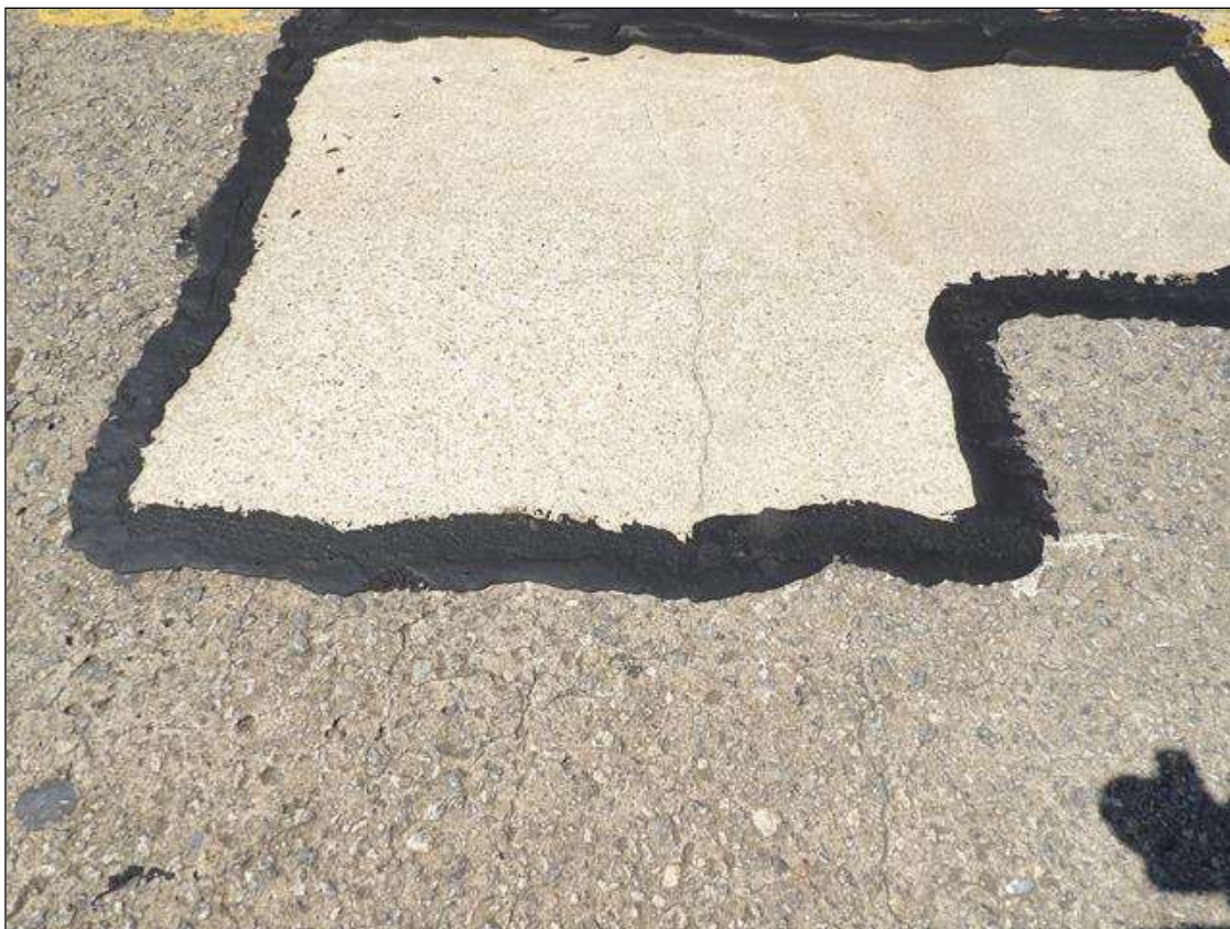
Span 4 Deck: SEVERAL SOUND DECK PATCHES UP TO 4.5 FEET X 3 FEET WITH CRACKING UP TO 1/32 INCHES WIDE
