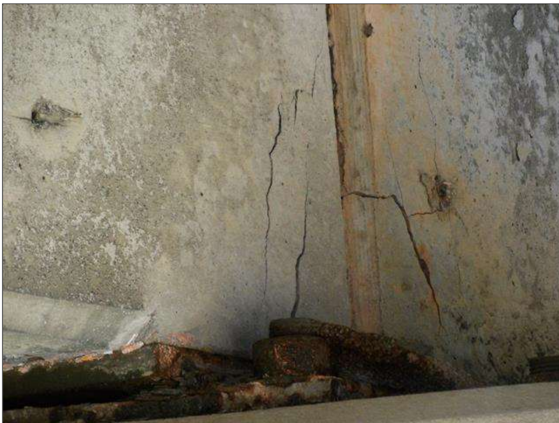
Span 4 Beam 4: AT BENT 3, 6 INCHES WIDE X 24 INCHES LONG DELAMINATION WITH CRACKING UP \frac{3}{32} INCHES WIDE ON LEFT SIDE AT END OF BEAM 4
