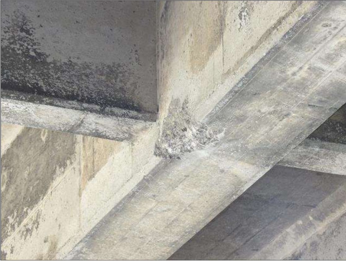
Span 2 Beam 3: IMPACT SPALL 15 INCHES LONG X 6 INCHES (BOTTOM FACE) X 6 INCHES (WEB) X 2 INCHES DEEP AT BOTTOM CORNER OF BEAM 3 NEAR MIDSPAN
