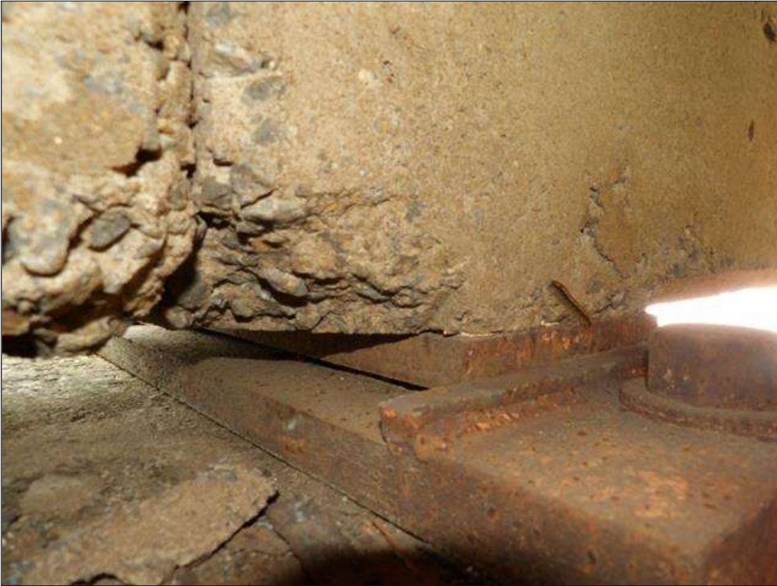
Span 2 Beam 1: 4 INCHES LONG X 3 INCHES WIDE X 1 1/2 INCHES DEEP SPALL ON BOTTOM RIGHT CORNER AT NEAR END, NO LOSS OF BEARING NOTED
