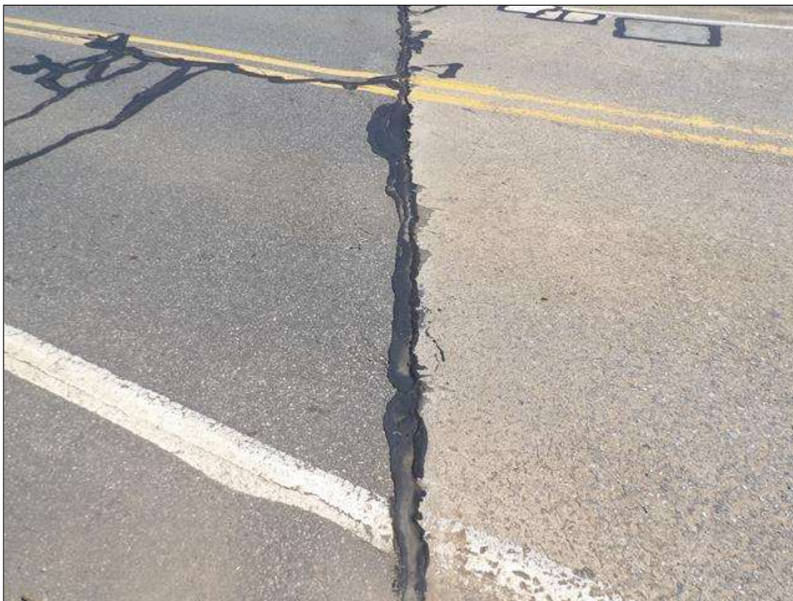
TYPICAL--JOINTS OVER SUBSTRUCTURES COVERED WITH TAR, JOINT OVER ABUTMENT 1 SHOWN
