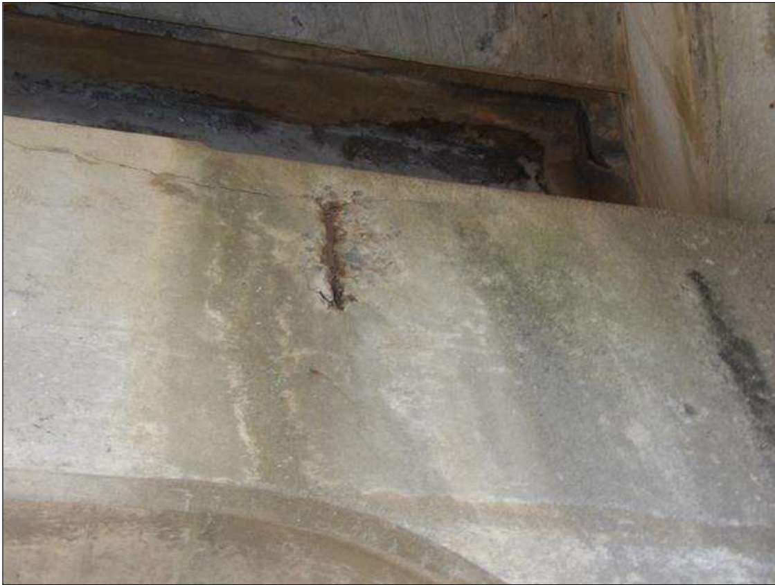
Bent 3 Cap 1: 18 INCHES HIGH X 8 INCHES WIDE X 1 INCHES DEEP SPALL WITH EXPOSED REBAR WITH ACTIVE CORROSION NO LOSS WITH A 3 FEET LONG HORIZONTAL CRACK UP TO 1/16 INCHES WIDE ON NEAR FACE OF CAP UNDER BAY 4
