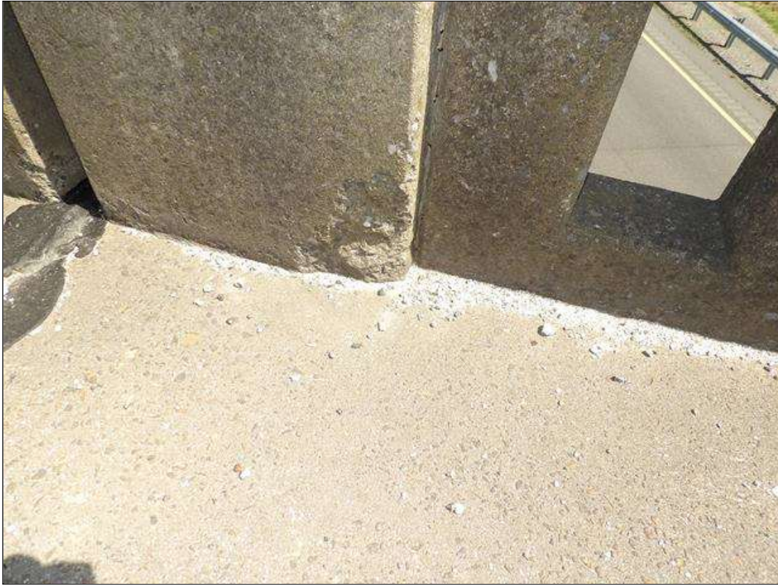
Span 3 Right Bridge Rail: SPALL 9 INCH X 6 INCH X 3/4 INCH DEEP ON INSIDE FACE OF END POSTS AT PIER 3 AT BOTTOM
