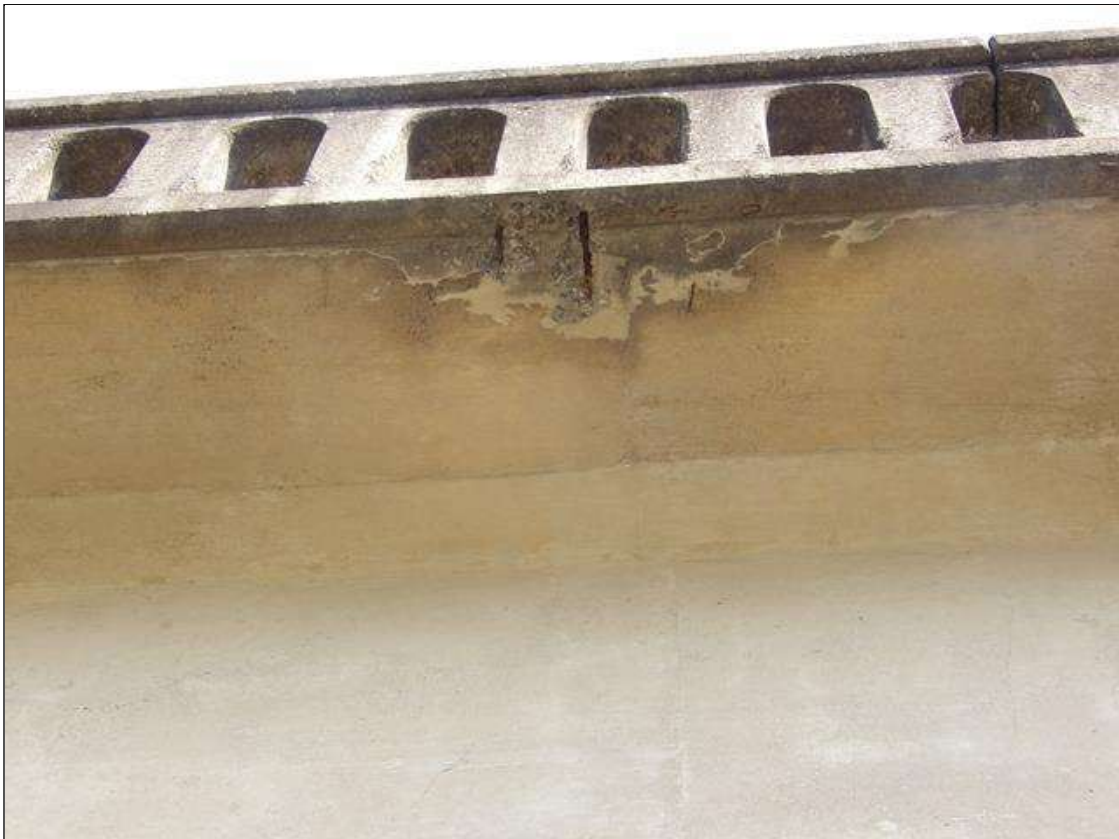
Span 2 Deck: 12 INCHES WIDE X 12 INCHES LONG X 1 INCHES DEEP SPALL WITH EXPOSED REBAR WITH ACTIVE CORROSION NO LOSS LOCATED AT UNDERSIDE OF LEFT OVERHANG 15 FEET FROM BENT 2
