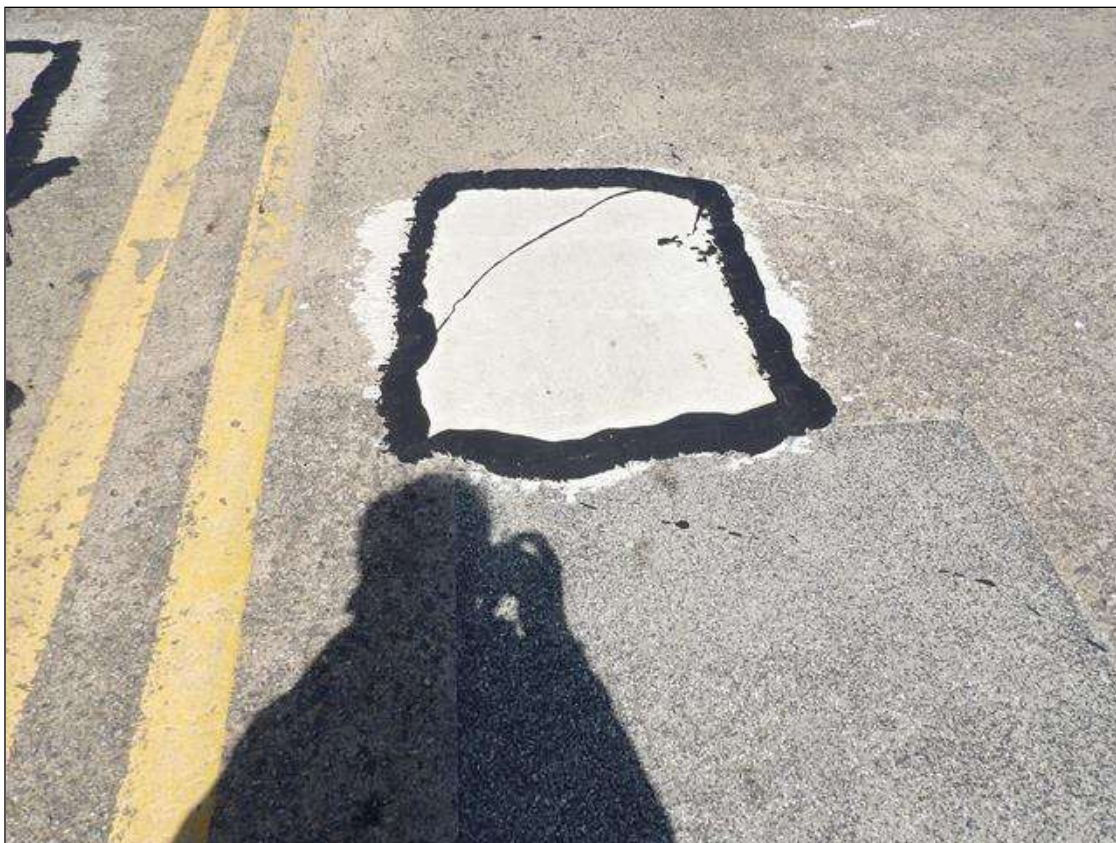
Span 1 Deck: SOUND PATCH 2 FEET DIAMETER IN NORTHBOUND LANE, APPROXIMATELY MIDSPAN
