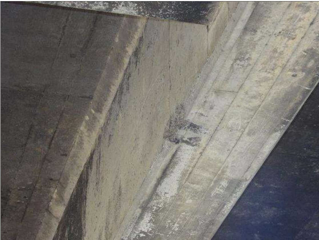
Span 2 Beam 4: IMPACT SPALL 8 INCHES LONG X 5 INCHES WIDE (BOTTOM FACE) X 3 INCHES HIGH (LEFT FACE) X 1 1/4 INCHES DEEP ON BOTTOM CORNER APPROXIMATELY MID-SPAN
