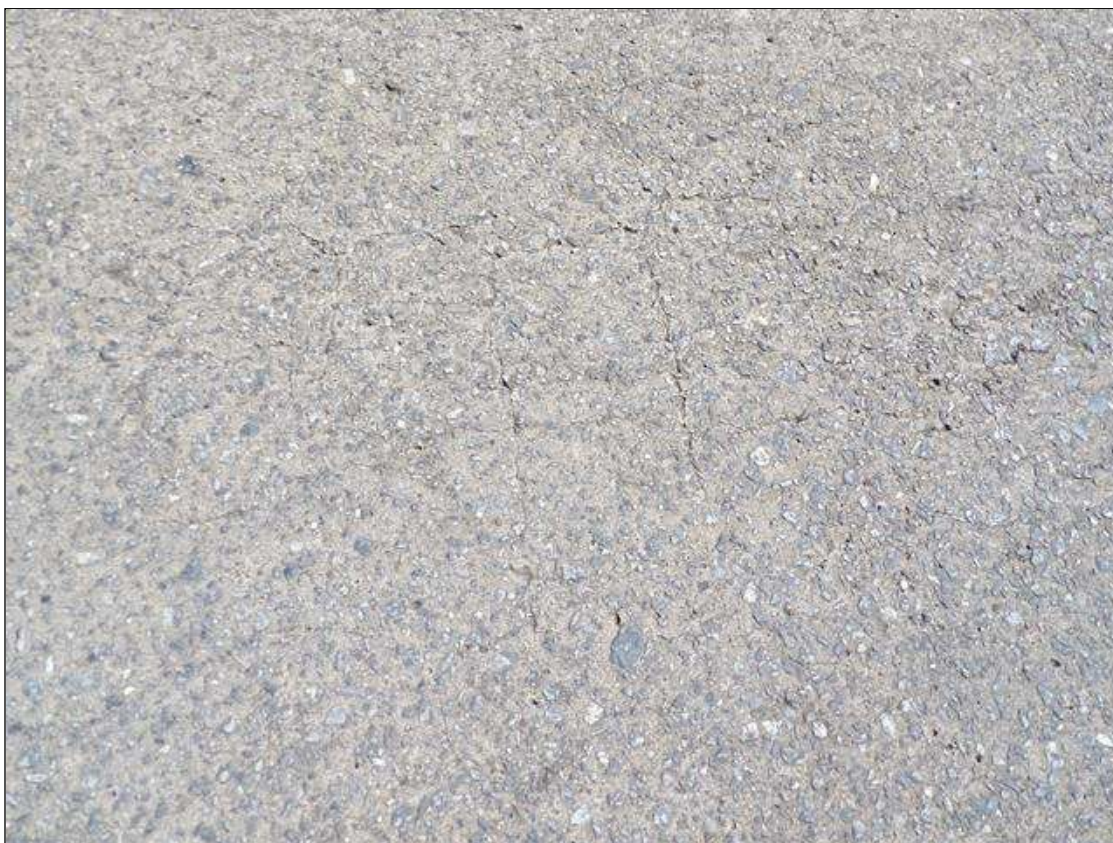
TYPICAL-- MAP CRACKING UP TO 1/16 INCHES WIDE INTERMITTENT THROUGHOUT BRIDGE DECK, SPAN 2 SHOWN
