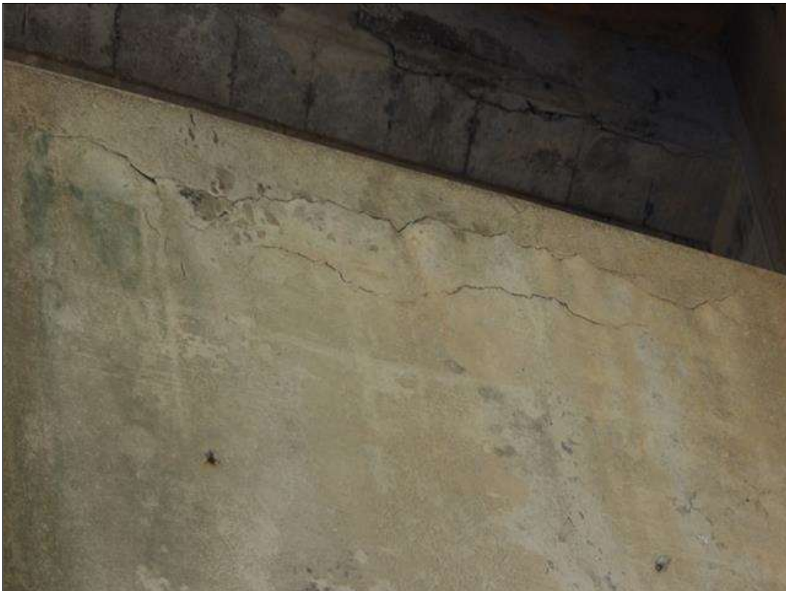
Bent 2 Cap 1: 4 FEET LONG X 10 INCHES HIGH DELAMINATION TOP OF FAR FACE WITH UP TO 1/8 INCHES WIDE CRACKING UNDER BAY 2
