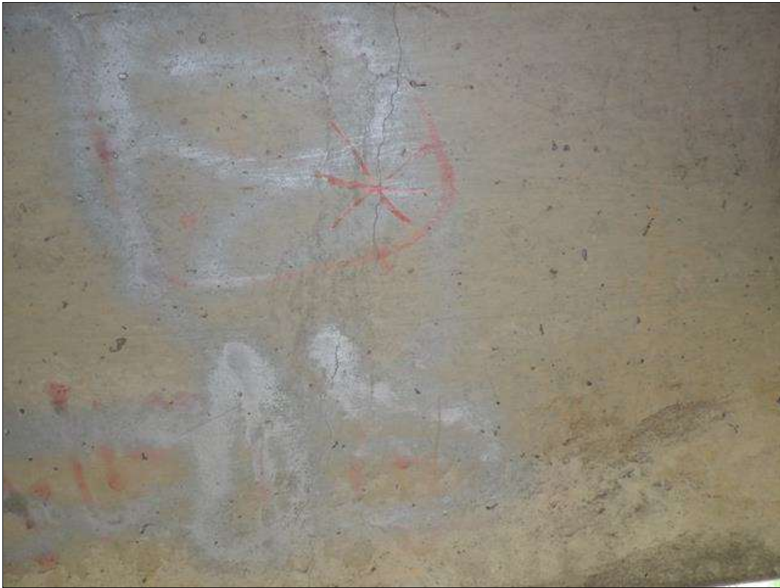
TYPICAL VERTICAL CRACKS UP TO 1/32 INCHES WIDE UP TO FULL-HEIGHT OF WEB SCATTERED THROUGHOUT BEAMS, BEAM 1 SPAN 1 SHOWN
