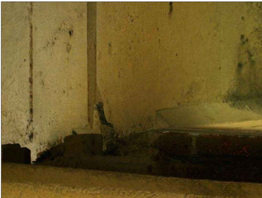
Span 4 Beam 3: AT BENT 3, DELAMINATION 4 INCHES HIGH X 4 INCHES WIDE ON END OF BEAM RIGHT CORNER
