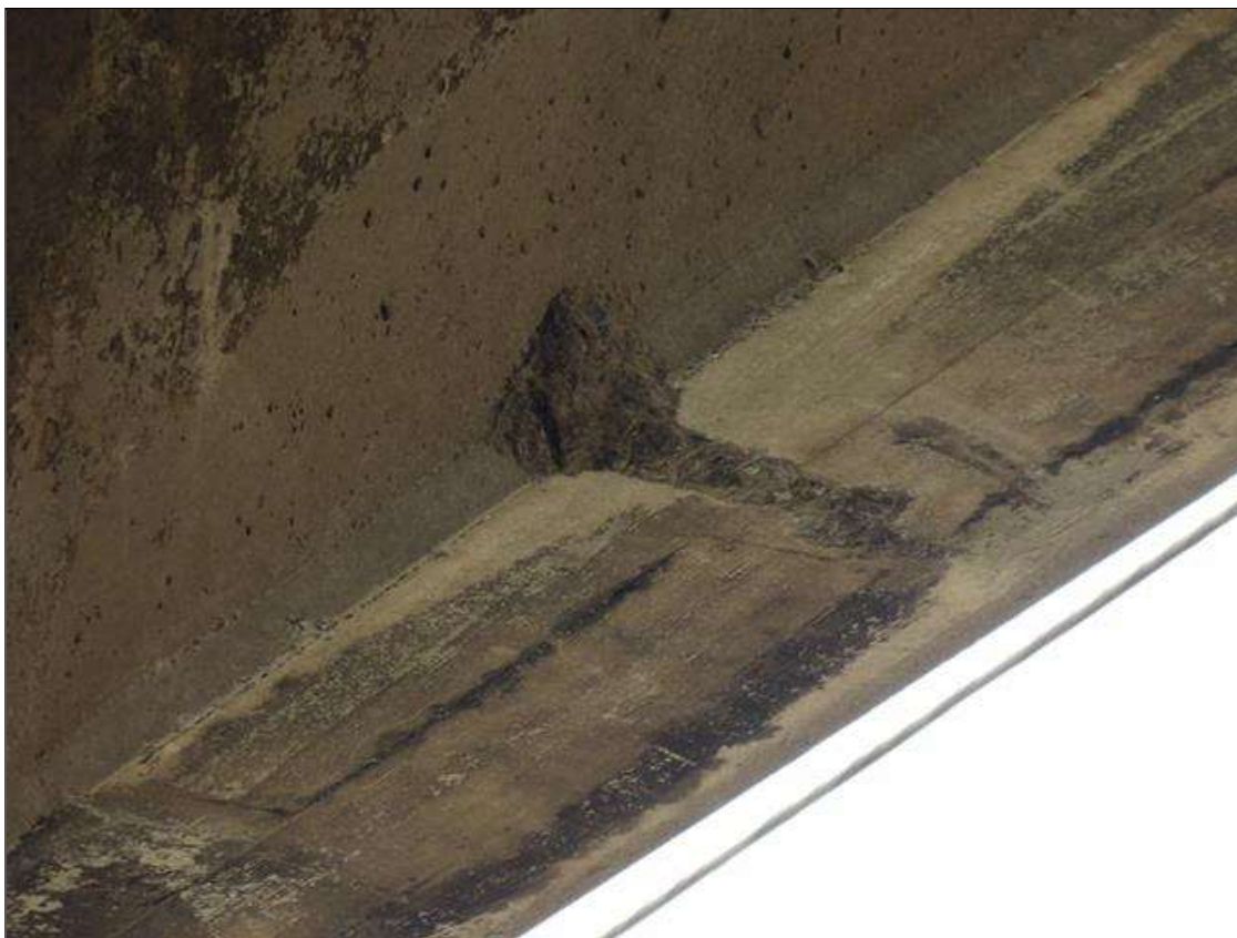
Span 2 Beam 5: IMPACT SPALL NEAR MIDSPAN, 6 INCHES X 4 INCHES X 2 INCHES DEEP AT BOTTOM OF BEAM
