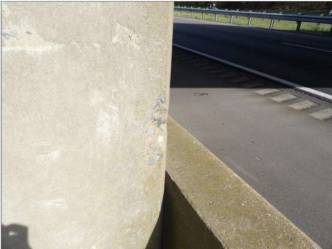
Bent 3 Pile 1: 6 INCHES X 3 INCHES X 1/2 INCHES DEEP SPALL WITH NO AT NEAR LEFT CORNER OF COLUMN 1 (BASE OF COLUMN)
