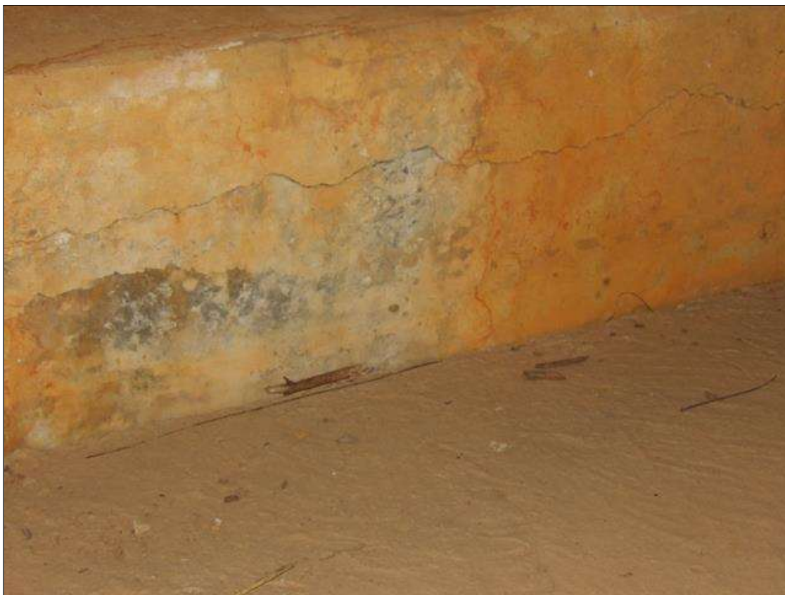
TYPICAL-- HORIZONTAL CRACK UP TO 1/16 INCHES WIDE ABUTMENT 2 CAP FACE, BAY 1 SHOWN
