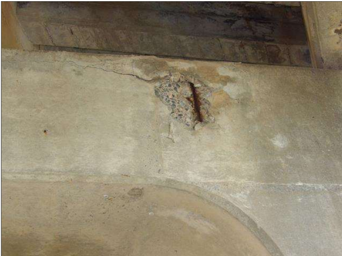
Bent 2 Cap 1: 4 FOOT-8 INCHES LONG X 1 FOOT-10 INCHES HIGH X 1 1/2 INCHES DEEP SPALL WITH EXPOSED REBAR/AREA OF DELAMINATION WITH ACTIVE CORROSION NO LOSS ON NEAR FACE IN BAY 4
