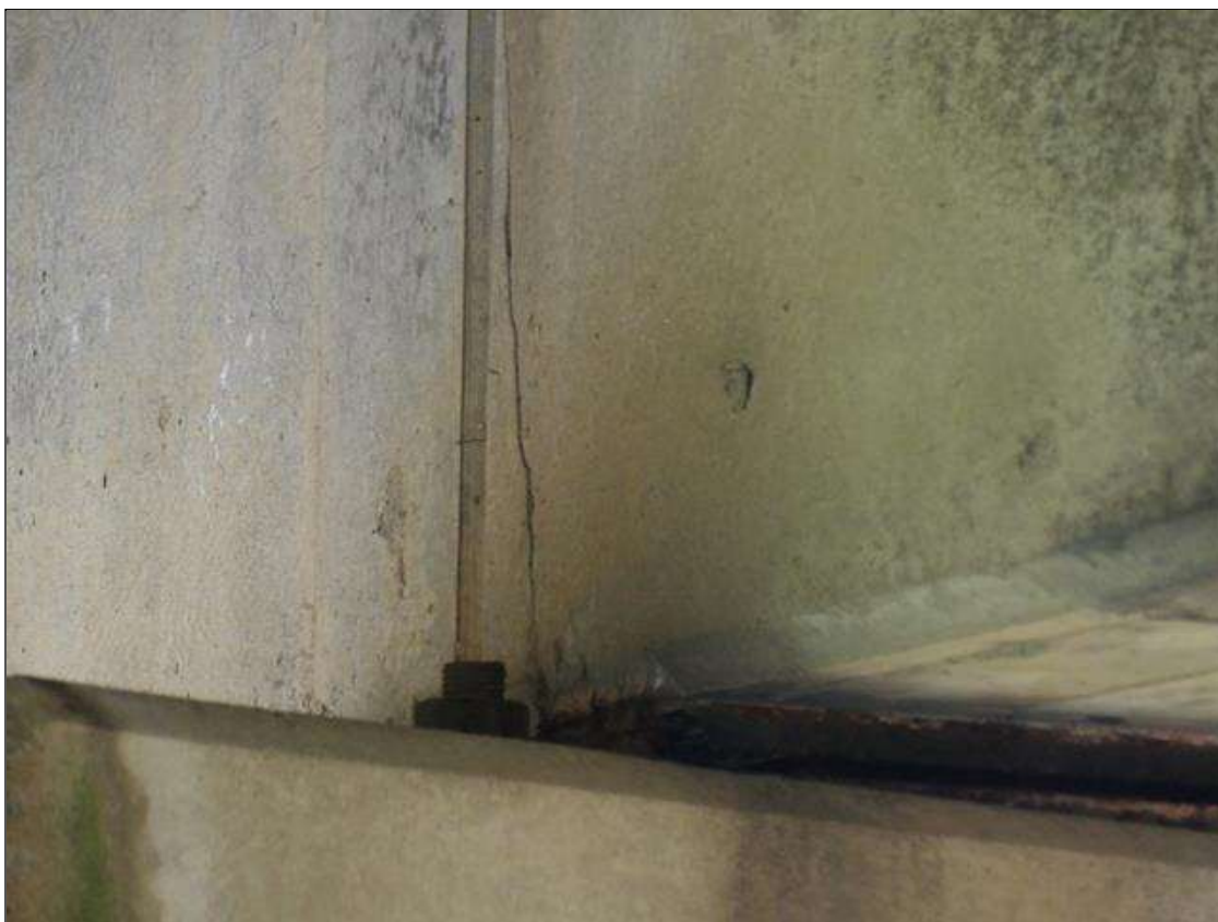
Span 4 Beam 4: 20 INCHES HIGH X 5 INCHES WIDE AREA OF DELAMINATION WITH UP TO \frac{1}{8} INCHES WIDE CRACKING ON RIGHT SIDE OF BEAM AT NEAR END
