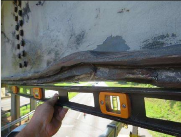
Crash damage on Bridge 110129 – 2021. Beam Out of Plumb.
