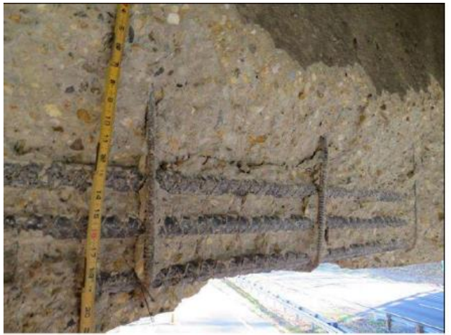
Crash Damage on Bridge 110106 – 11/23/21. Spalling with Exposed Rebar.
