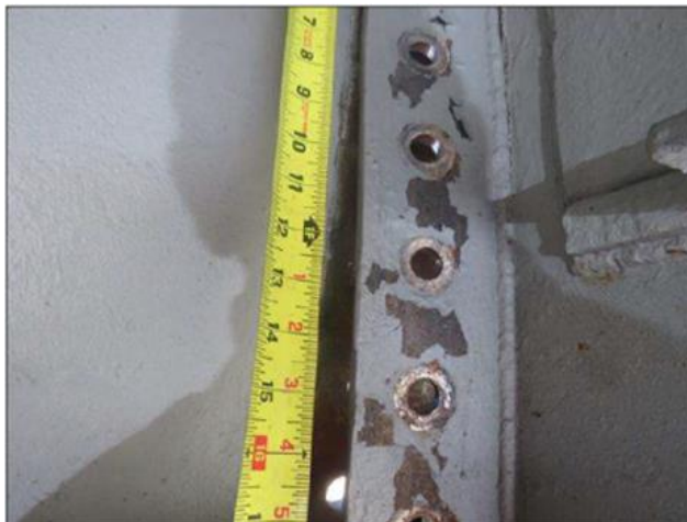
Crash damage on Bridge 110169 – 2023. Only 3 out of 10 bolts remained on the south side of Diaphragm 3.
