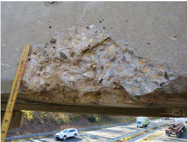
Crash Damage on Bridge 110106 – 11/23/24. Spalling.
