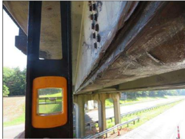
Crash damage on Bridge 110129 – 2021. Beam Out of Plumb.
