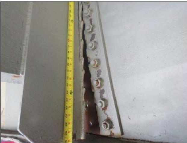
Crash damage on Bridge 110169 – 2023. The north side of the diaphragm is ripped loose.
