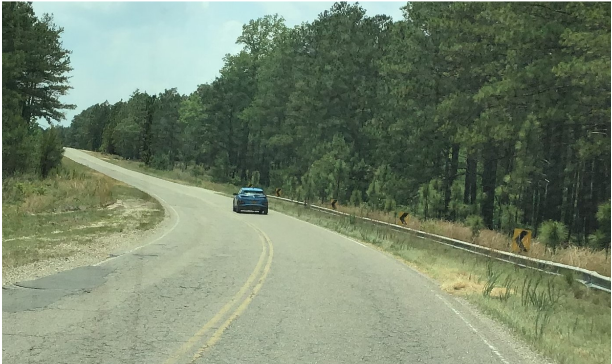
Guardrail proposed to be upgraded to current standard. Note terminal ends, and lack of blocks, and substandard height.
