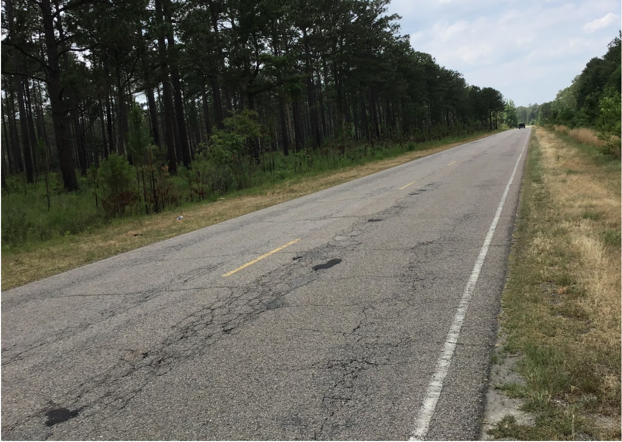
Picture indicating deteriorated pavement on Manchester Road
