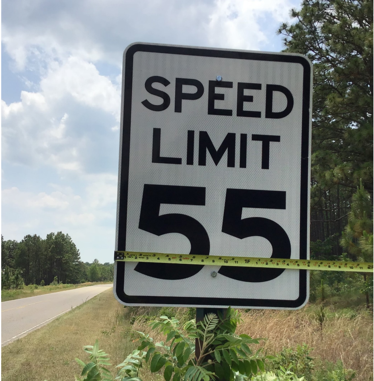
Existing Speed Limit signs 18"x24". Need to be upgraded to minimum of 24"x30"
