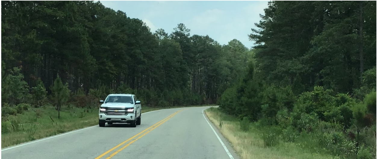
Vegetation growing in ditches, encroaching on shoulders within clear zone.
