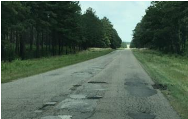
Figure 2 – Pavement Condition along King Road
