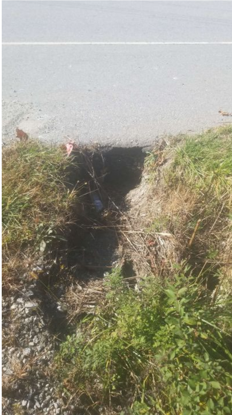
Image #2: Rill where it has reached the road
