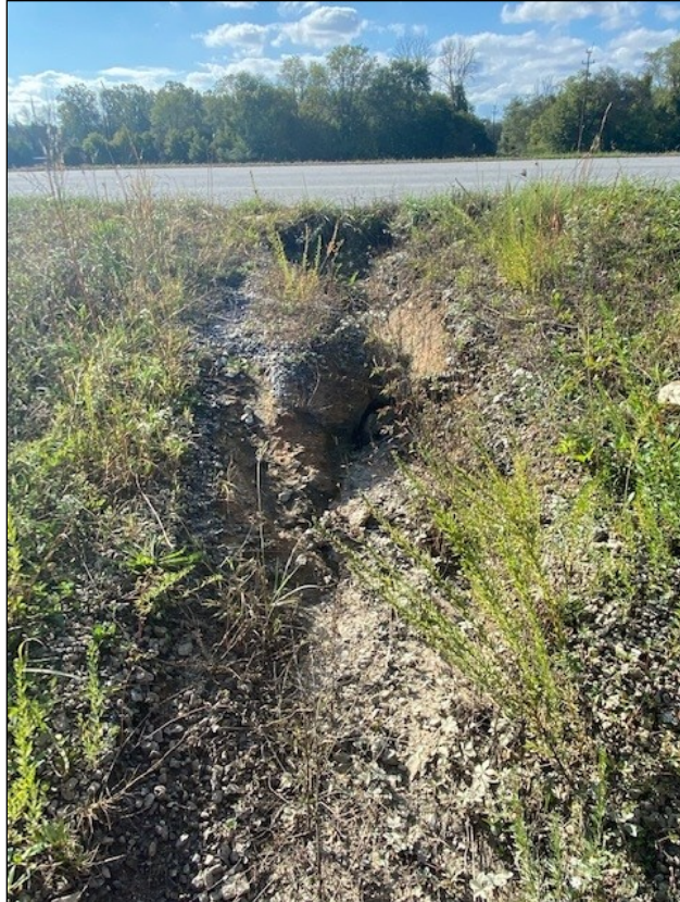
Photo 2 – Rill forming off Brookside Camp Road.
