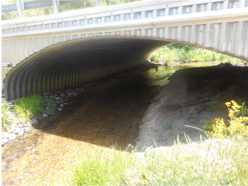
Figure 14. Native material backfilled over rip rap in aluminum box culvert (Henderson County, #440073, Greer Creek).
