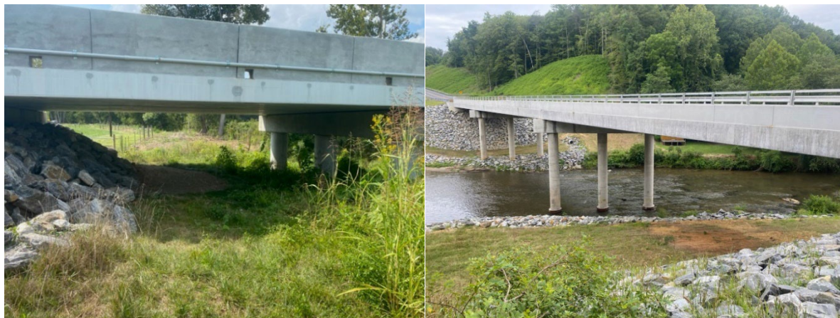
Figures 7 and 8. Unarmored floodplains under bridge in Iredell County (left, #480212, Patterson Creek) and large bridge in Stokes County (right, #840008, Dan River).
