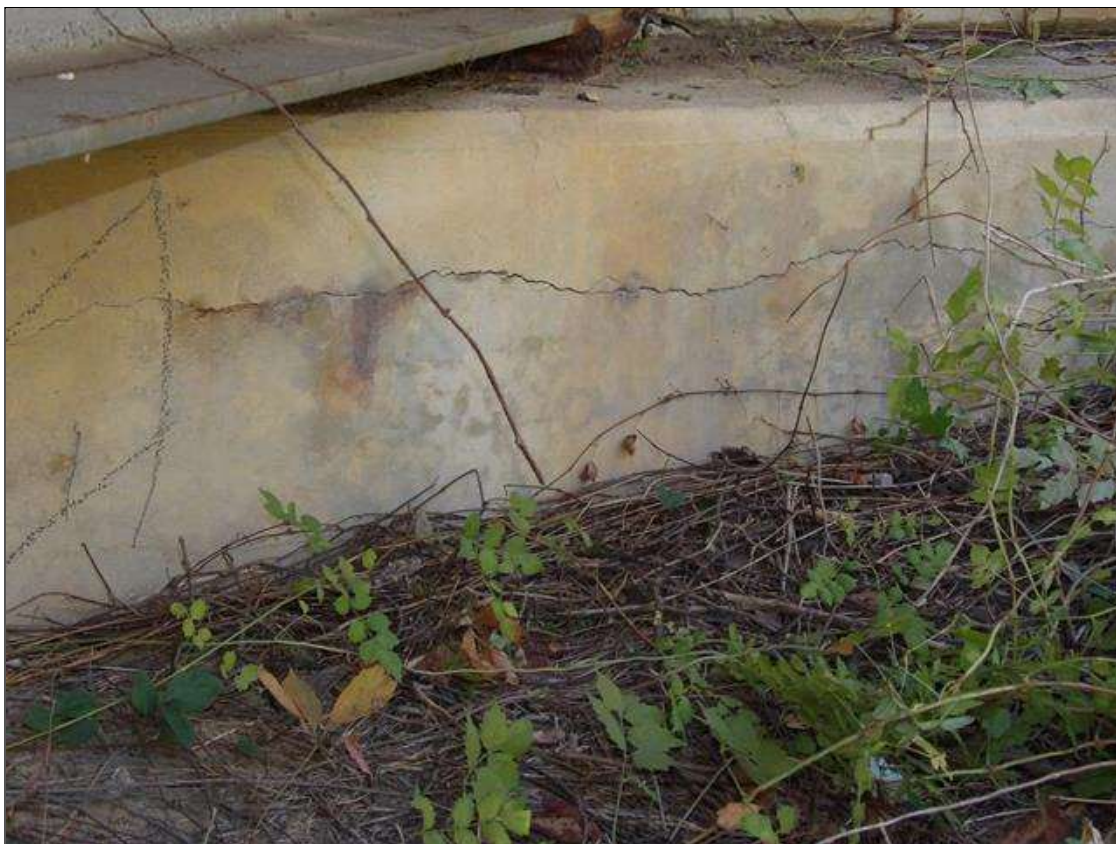
End Bent 1 Cap 1: 6 FEET HORIZONTAL CRACK UP TO 1/8 INCHES WIDE UNDER BEAM 1
