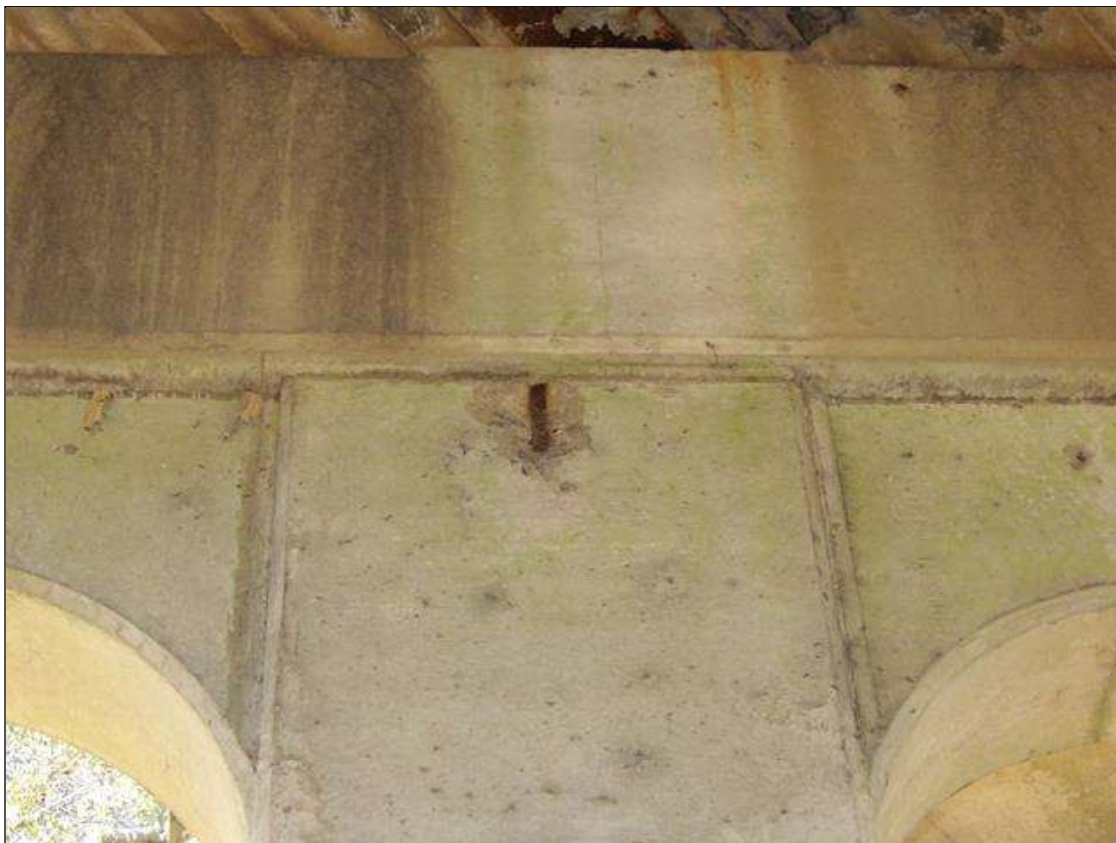
Bent 3 Pile 1: 9 INCHES X 6 INCHES X 1/2 INCHES DEEP SPALL WITH EXPOSED REBAR NO LOSS IN SOUTH FACE BELOW CAP
