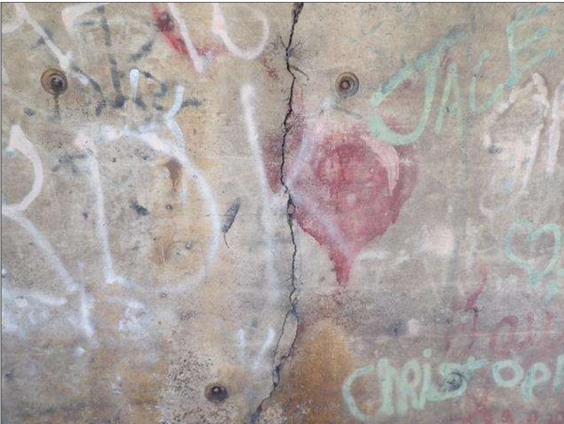
Bent 2 Pile 1: VERTICAL THRU CRACK 7 FOOT LONG UP TO 1/4 INCH WIDE WITH EDGE SPALLING IN MIDDLE OF CRASH WALL BOTH FACES
