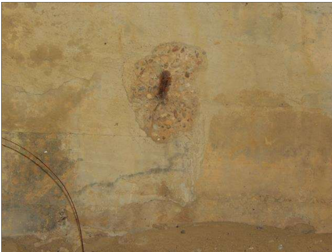
End Bent 1 Cap 1: 8 INCHES DIAMETER X 1 INCHES DEEP SPALL WITH EXPOSED REBAR NO LOSS UNDER BAY 4
