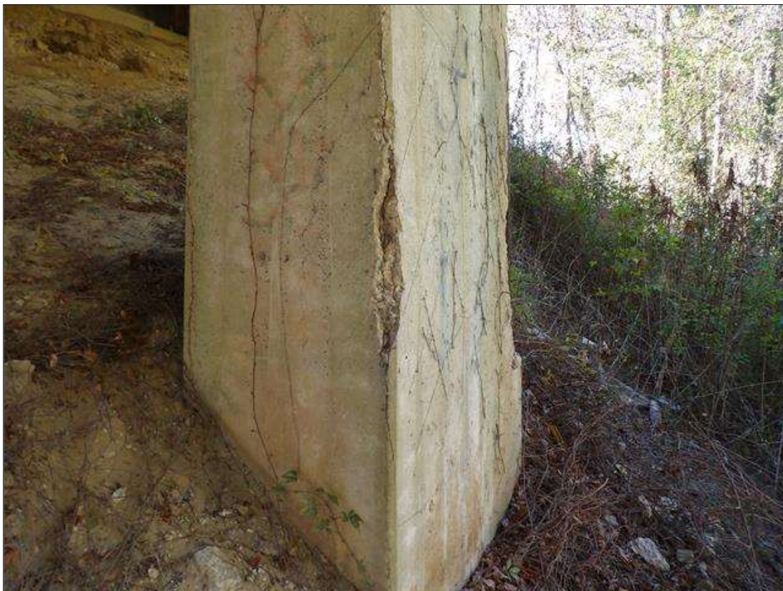
Bent 1 Pile 1: 24 FEET X 9 INCHES X 2 INCHES DEEP SPALL AND 5 FOOT X 3 FOOT DELAMINATION AT NORTHEAST CORNER
