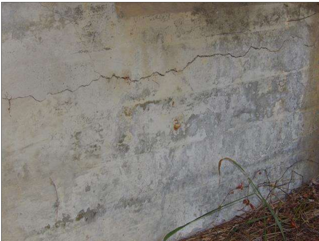
End Bent 2 Cap 1: HORIZONTAL CRACK 4 FEET LONG UP TO 1/8 INCH WIDE IN FACE OF CAP UNDER BEAM 5
