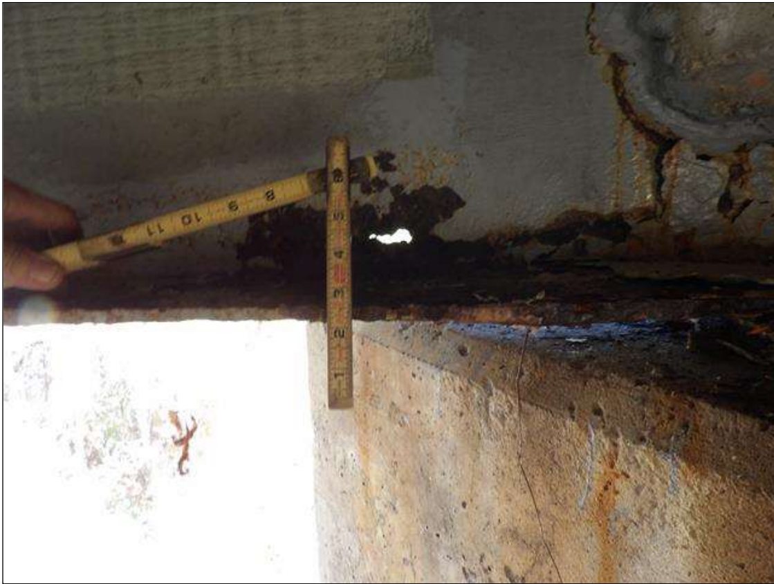
Span 5 Beam 5: PAR--BEAM END AT BENT 4 IN THE LOWER FLANGE, CORROSION WITH SECTION LOSS [AVERAGE 1/4 INCHES AVERAGE REMAINS FULL WIDTH] FOR APPROXIMATELY 4 FEET LONG. AT THE SAME END IN THE LOWER 4 INCHES OF THE WEB, CORROSION WITH 100 PERCENT SECTION LOSS WITH 1 INCH X 1/2 INCH HOLE 2 FEET FROM BEAM END [AVERAGE 5/16 INCHES REMAINS] FOR APPROXIMATELY 4 FEET LONG.
