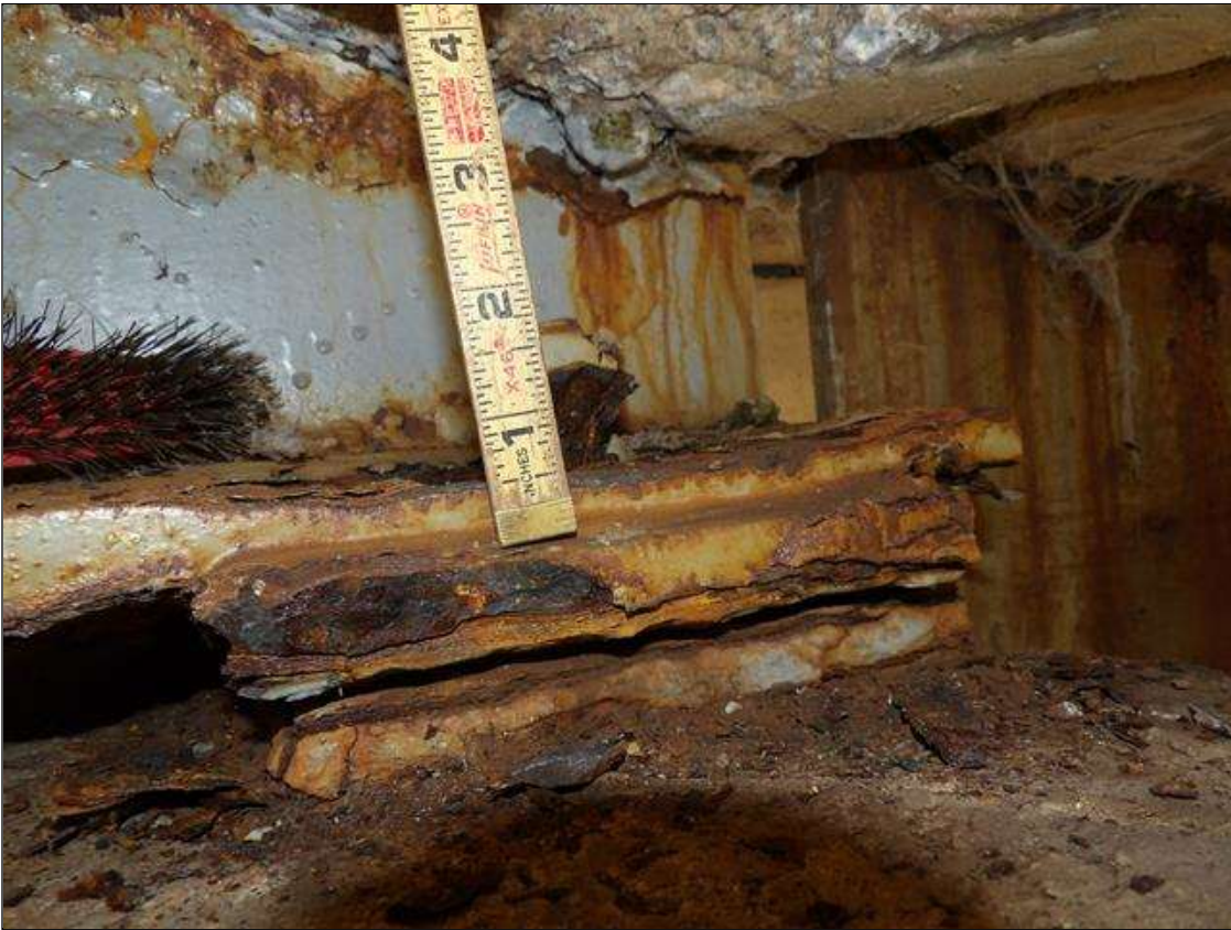
Span 4 Beam 2: PAR--SECTION LOSS IN BOTTOM FLANGE UP TO 1/4 INCHES WITH 1/2 INCHES AVERAGE REMAINING FULL WIDTH 9 INCHES LONG AT BEAM END OVER PIER 3.
