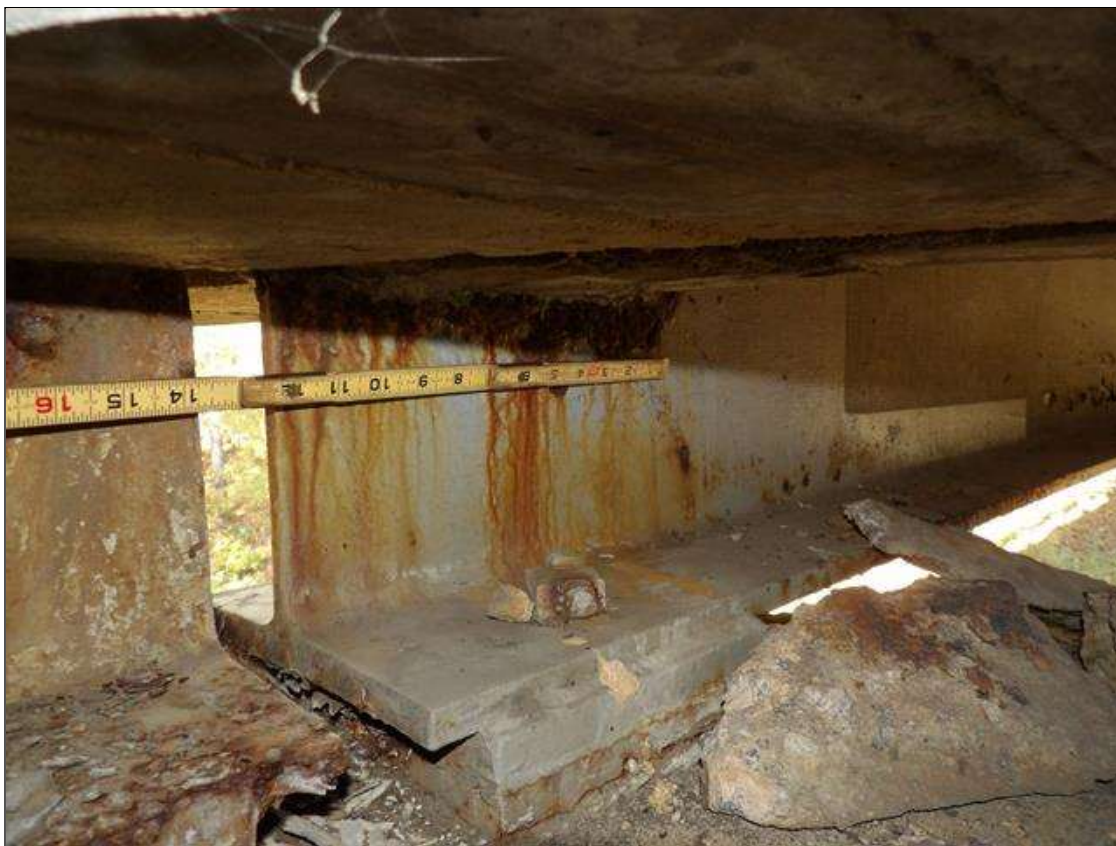
Span 2 Beam 1: PAR--BEAM END AT BENT 1 AT THE INTERFACE WITH THE REINFORCED CONCRETE DIAPHRAGM, THERE IS A BAND OF CORROSION UP TO 2 INCHES WIDE WITH SECTION LOSS [AVERAGE 3/8 INCHES REMAINS] FOR APPROXIMATELY 1 FEET LONG X UP TO THE FULL HEIGHT OF THE DIAPHRAGM.
