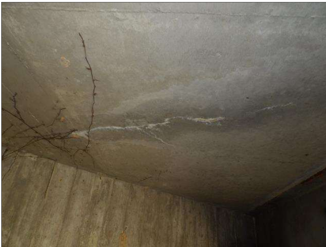
Span 5 Deck: 7 FEET LONG HAIRLINE DIAGONAL CRACK WITH MINOR EFFLORESCENCE IN UNDERSIDE OF DECK BAY 4 AT ABUTMENT 2
