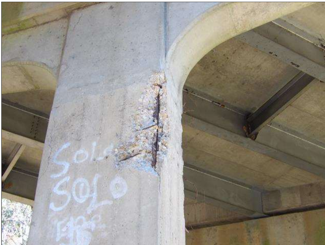
Bent 3 Pile 2: PAR--SOUTHEAST CORNER, SPALLING WITH EXPOSED REBAR [APPROXIMATELY 4 FEET HIGH X UP TO 1.25 FEET WIDE X UP TO 3 INCHES DEEP]
