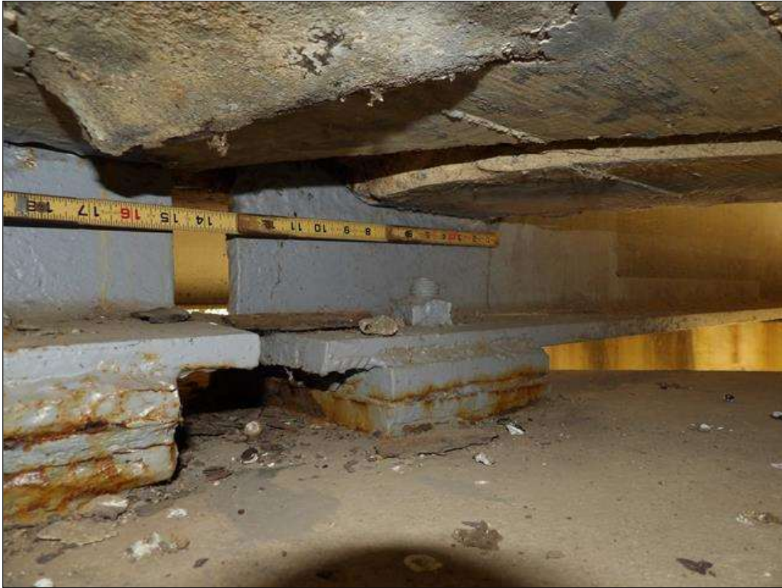
Span 4 Beam 3: PAR--BEAM END AT BENT 4 AT THE INTERFACE WITH THE REINFORCED CONCRETE DIAPHRAGM, THERE IS A BAND OF CORROSION UP TO 1 INCHES WIDE WITH SECTION LOSS [AVERAGE 5/16 INCHES REMAINS] FOR APPROXIMATELY 1 FEET LONG X UP TO THE FULL HEIGHT OF THE DIAPHRAGM. BEAM END HAS BEEN PAINTED WITH NO ACTIVE CORROSION
