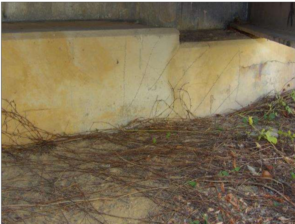
End Bent 1 Cap 1: DELAMINATION 3 FEET LONG X 2 FEET HIGH UNDER BEAM 1 NORTH FACE
