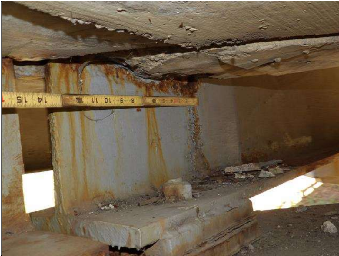
Span 2 Beam 2: PAR--BEAM END AT BENT 1 AT THE INTERFACE WITH THE REINFORCED CONCRETE DIAPHRAGM, THERE IS A BAND OF CORROSION UP TO 3 INCHES WIDE WITH SECTION LOSS [AVERAGE 3/8 INCHES REMAINS] FOR APPROXIMATELY 1 FOOT LONG X UP TO THE FULL HEIGHT OF THE DIAPHRAGM.
