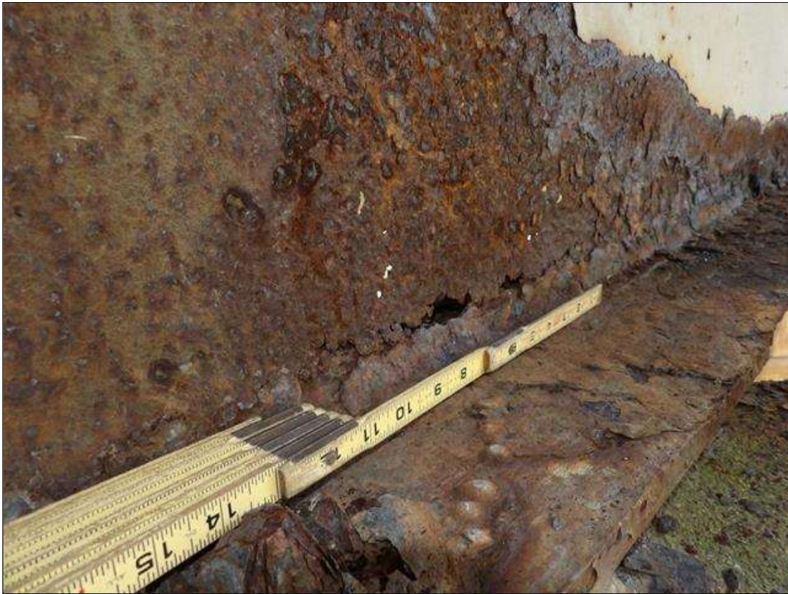
Span 3 Beam 1: PAR-- BEAM END AT BENT 3 IN THE LEFT LOWER FLANGE, CORROSION WITH SECTION LOSS DOWN TO KNIFE EDGE [AVERAGE 3/8 INCHES REMAINS FULL WIDTH OF FLANGE ] FOR APPROXIMATELY 4 FEET LONG WITH EDGE HOLES UP TO 3/4 INCHES DIAMETER. AT THE SAME END IN THE LOWER 6 INCHES OF THE WEB, CORROSION WITH SECTION LOSS [AVERAGE 1/16 INCHES REMAINS] FOR APPROXIMATELY 4 FEET LONG WITH PERFORATIONS THROUGHOUT.
