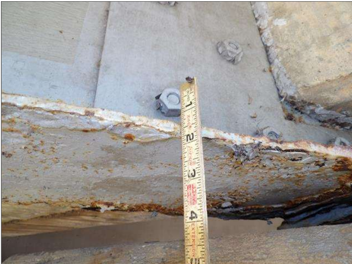
Span 4 Beam 1: PAR--BEAM END AT BENT 3 IN THE LOWER FLANGE, CORROSION WITH SECTION LOSS [AVERAGE 3/8 INCHES REMAINS FULL WIDTH OF FLANGE] FOR APPROXIMATELY 3 FEET LONG.
