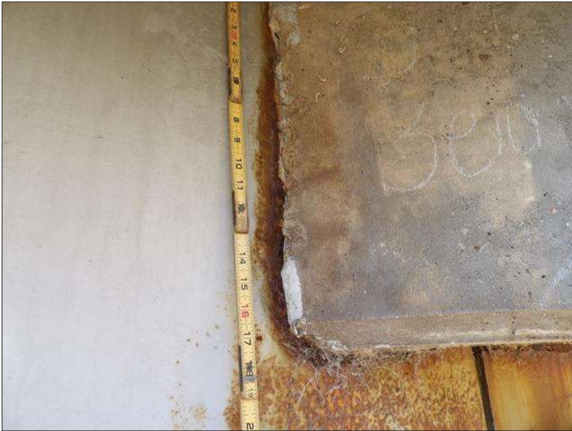
Span 1 Beam 5: PAR--BEAM END AT BENT 1 AT THE INTERFACE WITH THE REINFORCED CONCRETE DIAPHRAGM, THERE IS A BAND OF CORROSION UP TO 2 INCHES WIDE WITH SECTION LOSS [AVERAGE 3/16 INCHES REMAINS] FOR APPROXIMATELY 1 FEET LONG X UP TO THE FULL HEIGHT OF THE DIAPHRAGM.
