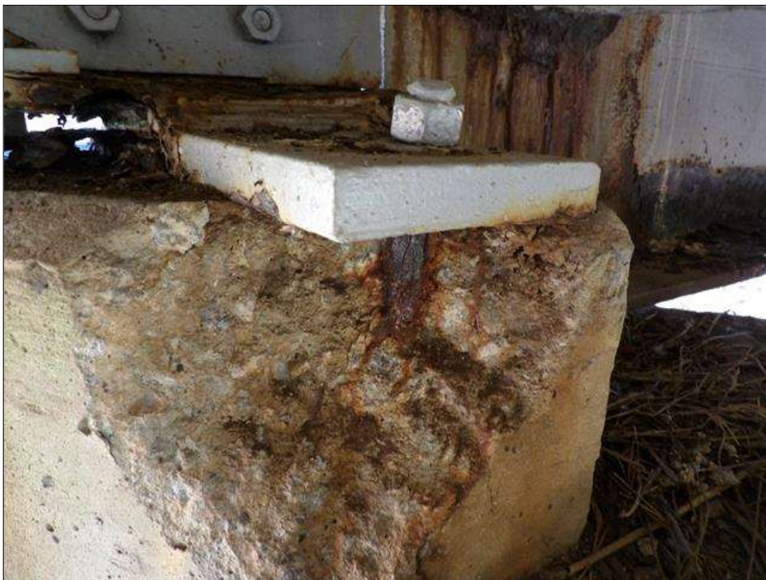
Span 4 Near Bearing 5: PAR--BEARING LATERAL RETROFIT PLATE ON LEFT SIDE OF BEARING WITH EXPOSED BENT ANCHOR BOLT DUE TO SPALL IN CAP
