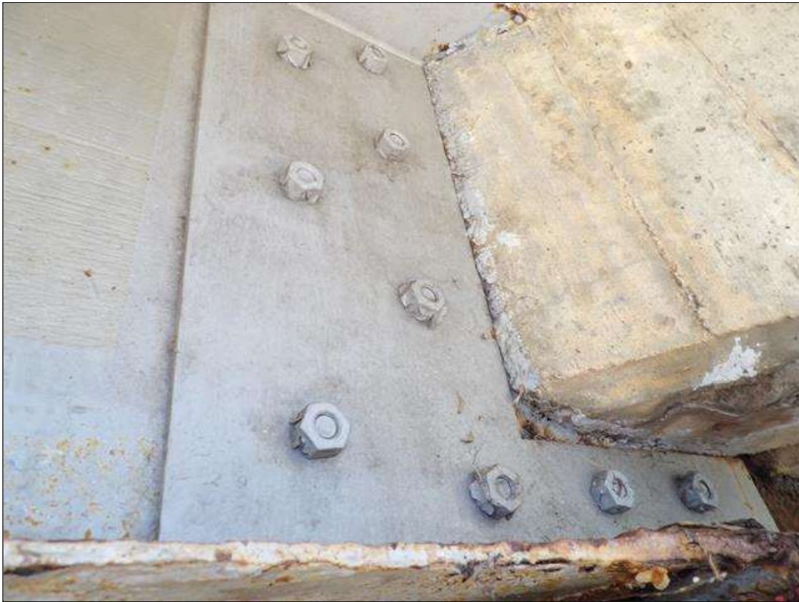
SPAN 4 BEAM 1 BOLTED PLATE REPAIR FULL HEIGHT X 1 FOOT LONG TO WEB AT BENT 3, BEAMS 3 AND 5 SIMILAR
