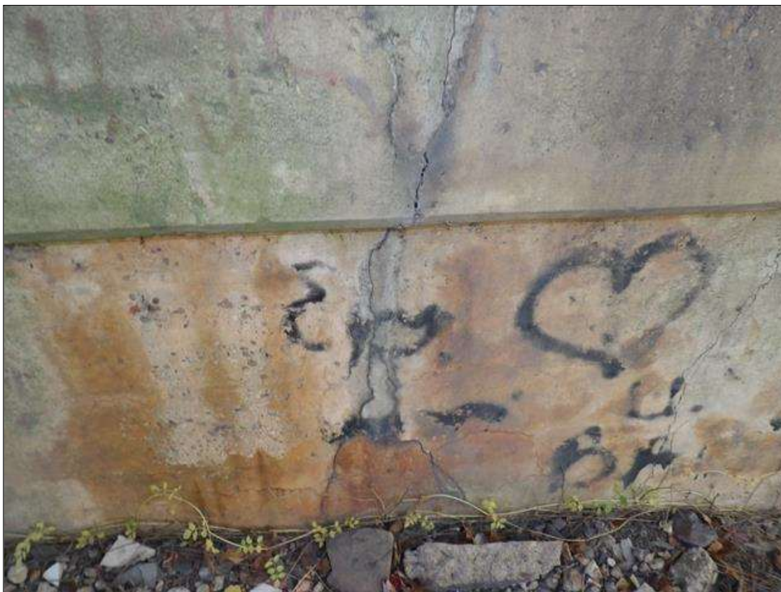
Bent 3 Pile 1: VERTICAL THROUGH CRACK 7 FOOT LONG X 1/8 INCHES WIDE IN MIDDLE OF CRASHWALL BOTH FACES
