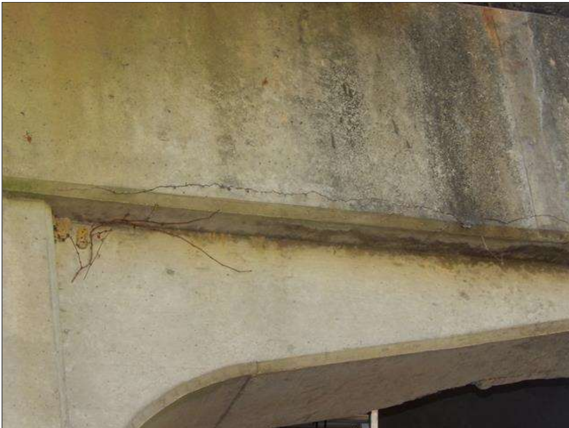
Bent 1 Cap 1: 6 FEET LONG X 1/8 INCHES WIDE HORIZONTAL CRACK NORTH FACE UNDER BAY 1 AND A 1/16 INCH WIDE HORIZONTAL CRACK 1.5 FOOT LONG UNDER BEAM 4
