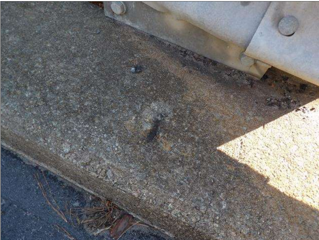
Span 1 Right Bridge Rail: 3 INCHES X 1 INCHES X 1/2 INCHES DEEP SPALL WITH EXPOSED REBAR NO LOSS IN TOP OF CURB AT GUARDRAIL ATTACHMENT
