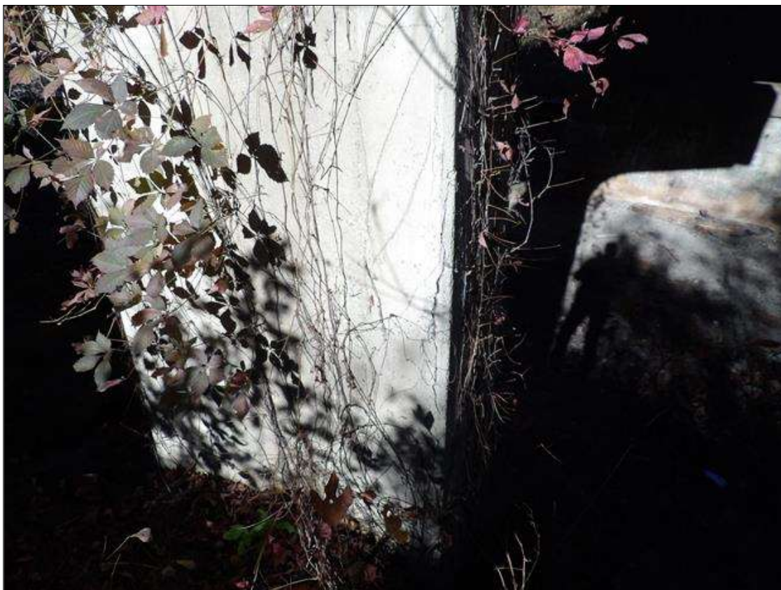
Bent 1 Pile 2: 6 FOOT X 1.5 FOOT AREA OF DELAMINATION ON SOUTHEAST CORNER
