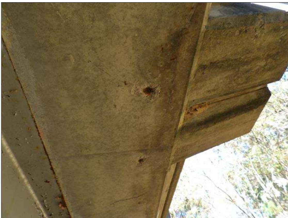
TYPICAL--SPALL WITH EXPOSED REBAR NO LOSS IN EAST/WEST EDGES OF DECK 4 INCHES DIAMETER X 1 INCHES DEEP IN SPAN 5 DECK
