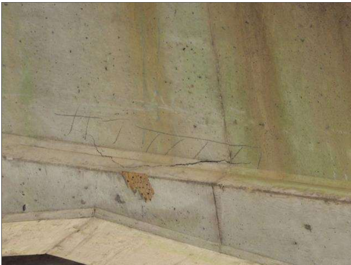
Bent 2 Cap 1: 3 FEET X 1.5 FEET HIGH DELAMINATION IN SOUTH FACE UNDER BEAM 3
