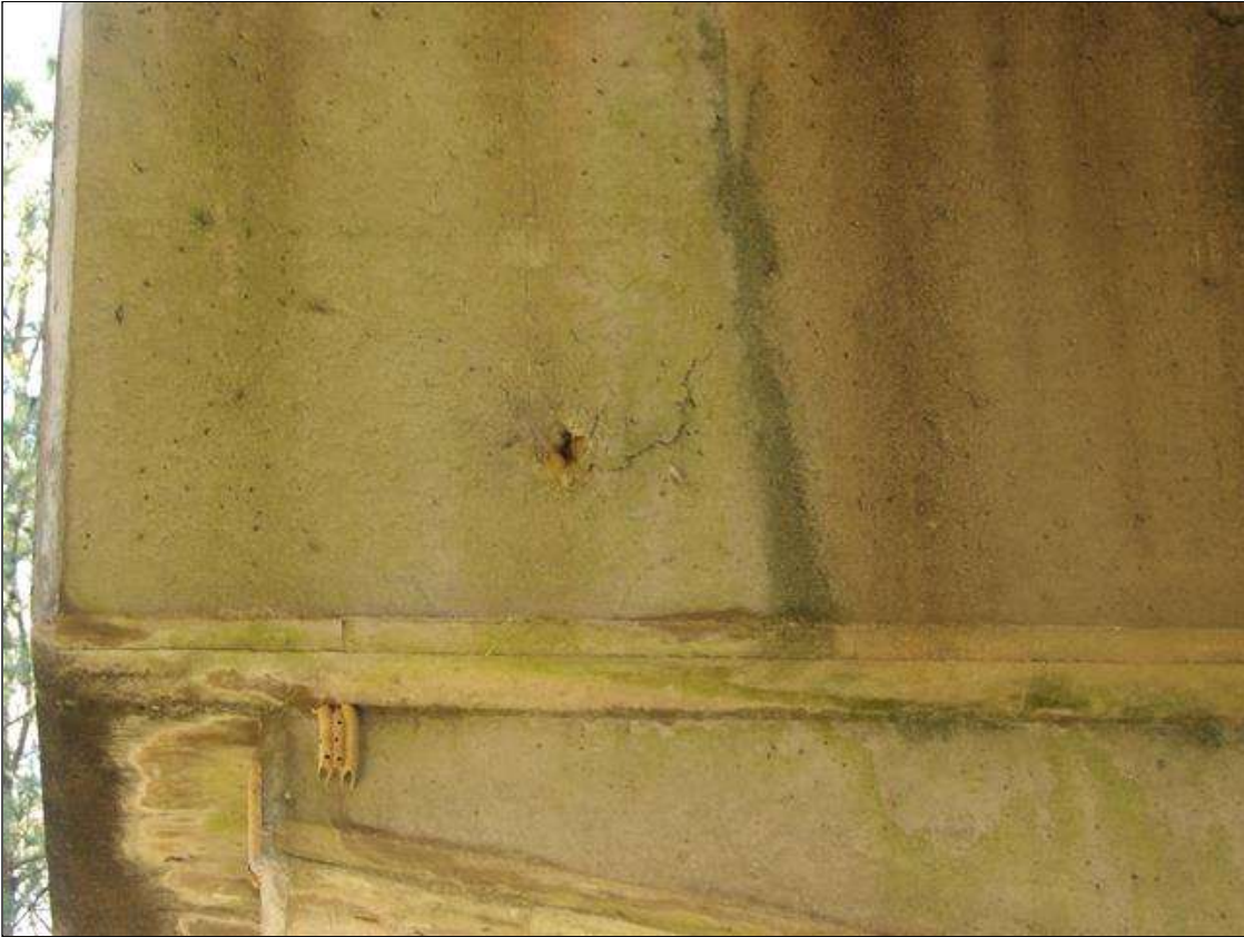
Bent 3 Cap 1: 9 INCHES DIAMETER DELAMINATION WITH SPALL 3 INCH X 2 INCH X 1 INCH DEEP WITH EXPOSED REBAR NO LOSS NORTH FACE UNDER BEAM 5
