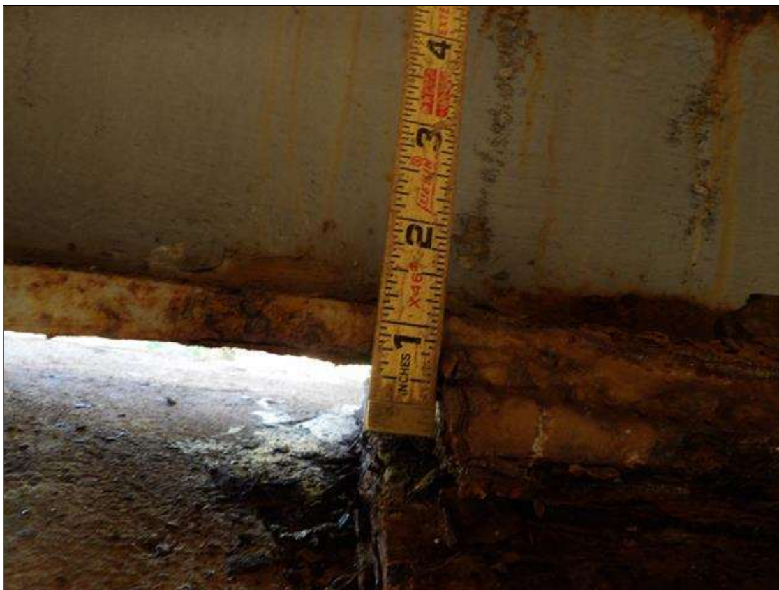
Span 2 Beam 1: 1 FEET OF CORROSION WITH 1/2 INCHES REMAINING SECTION IN BOTTOM FLANGE AND 7/16 INCHES REMAINING SECTION IN WEB AROUND END DIAPHRAGM AT BENT 2 HAS BEEN PREVIOUSLY PAINTED OVER WITH ACTIVE CORROSION.
