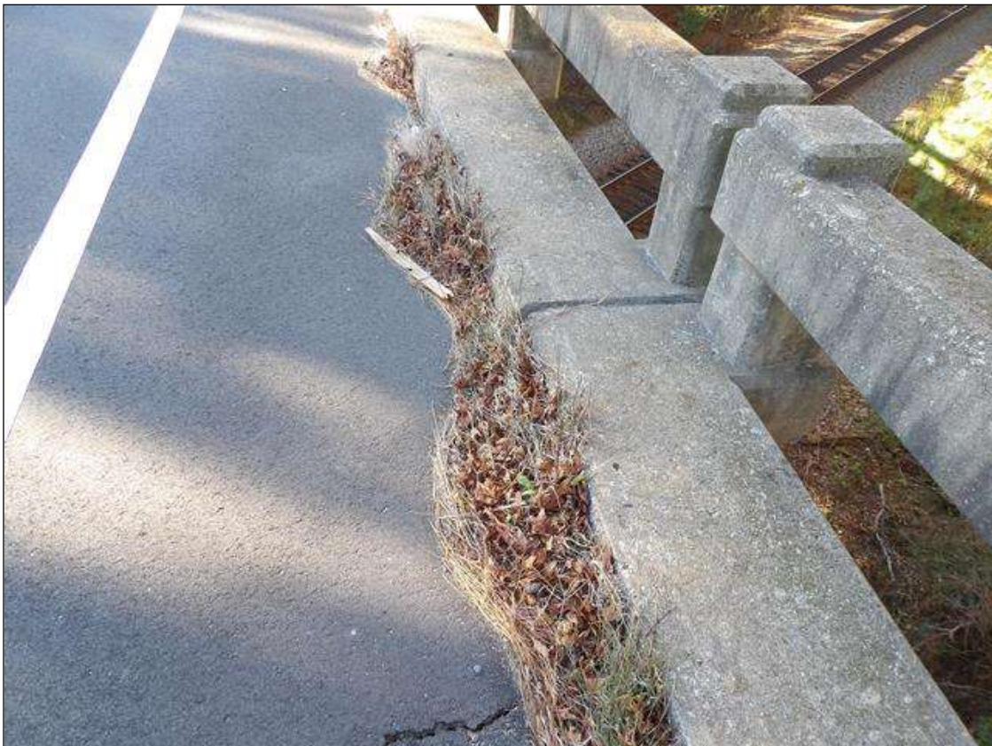
MINOR DEBRIS ACCUMULATION ALONG LEFT RAIL
