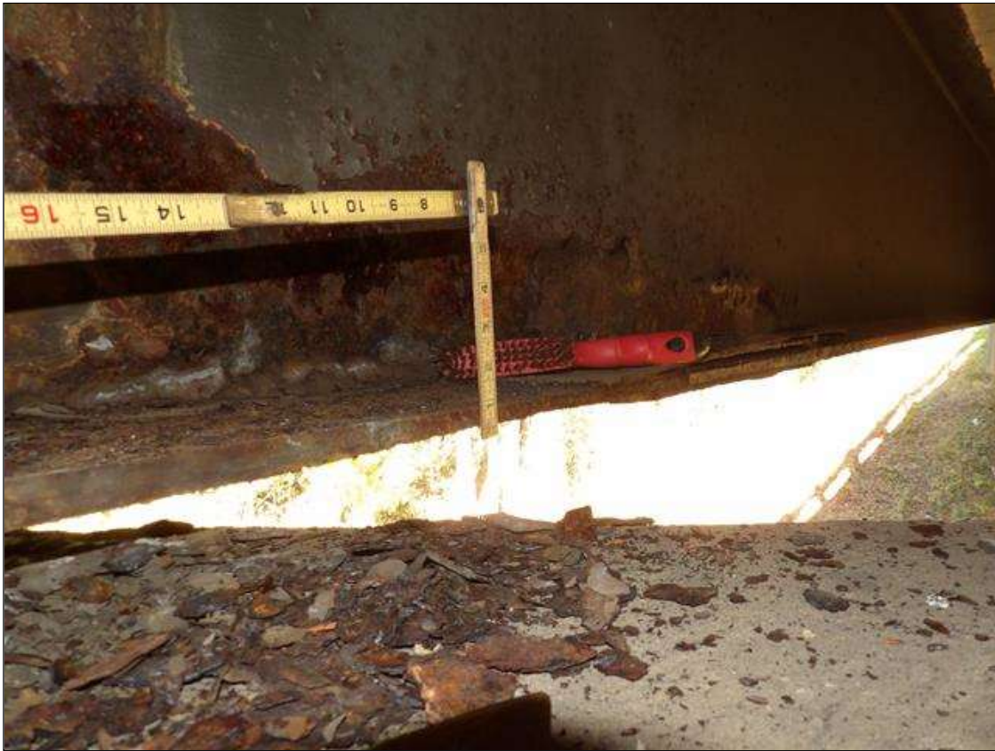
Span 3 Beam 1: PAR--CORROSION AROUND DIAPHRAGM OVER PIER 2- 2 INCHES WIDE WITH 3/8 INCHES AVERAGE REMAINING THICKNESS AND 6 INCHES HIGH IN BOTTOM OF WEB 4 FEET LONG. CORROSION IN BOTTOM FLANGE 4 FOOT LONG WITH 7/16 INCH SECTION LOSS WITH 1/2 INCH AVERAGE REMAINING STARTING AT PIER 2
