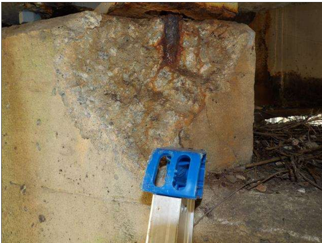
Bent 3 Cap 1: SPALL 9 INCH X 9 INCH X 3 INCHES DEEP WITH EXPOSED REBAR NO LOSS IN PEDESTAL AT BEAM 5 NORTH FACE. PAR SENT UNDER BEARING
