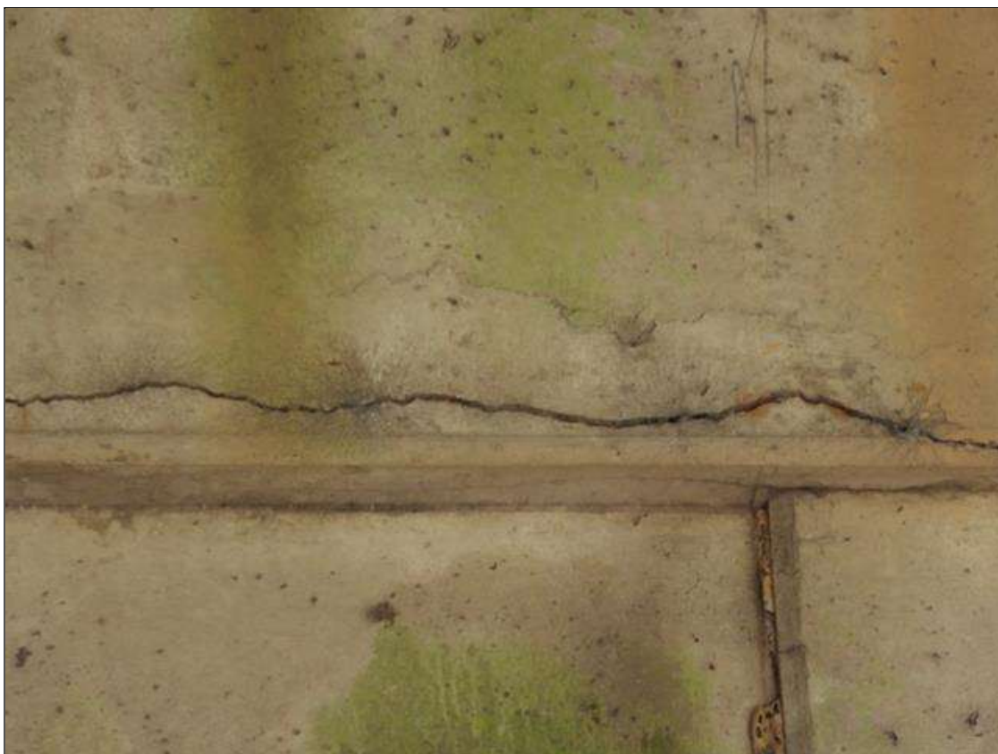
Bent 2 Cap 1: 6 FEET LONG HORIZONTAL CRACK UP TO 1/4 INCHES WIDE UNDER BAYS 1 AND 2 NORTH FACE
