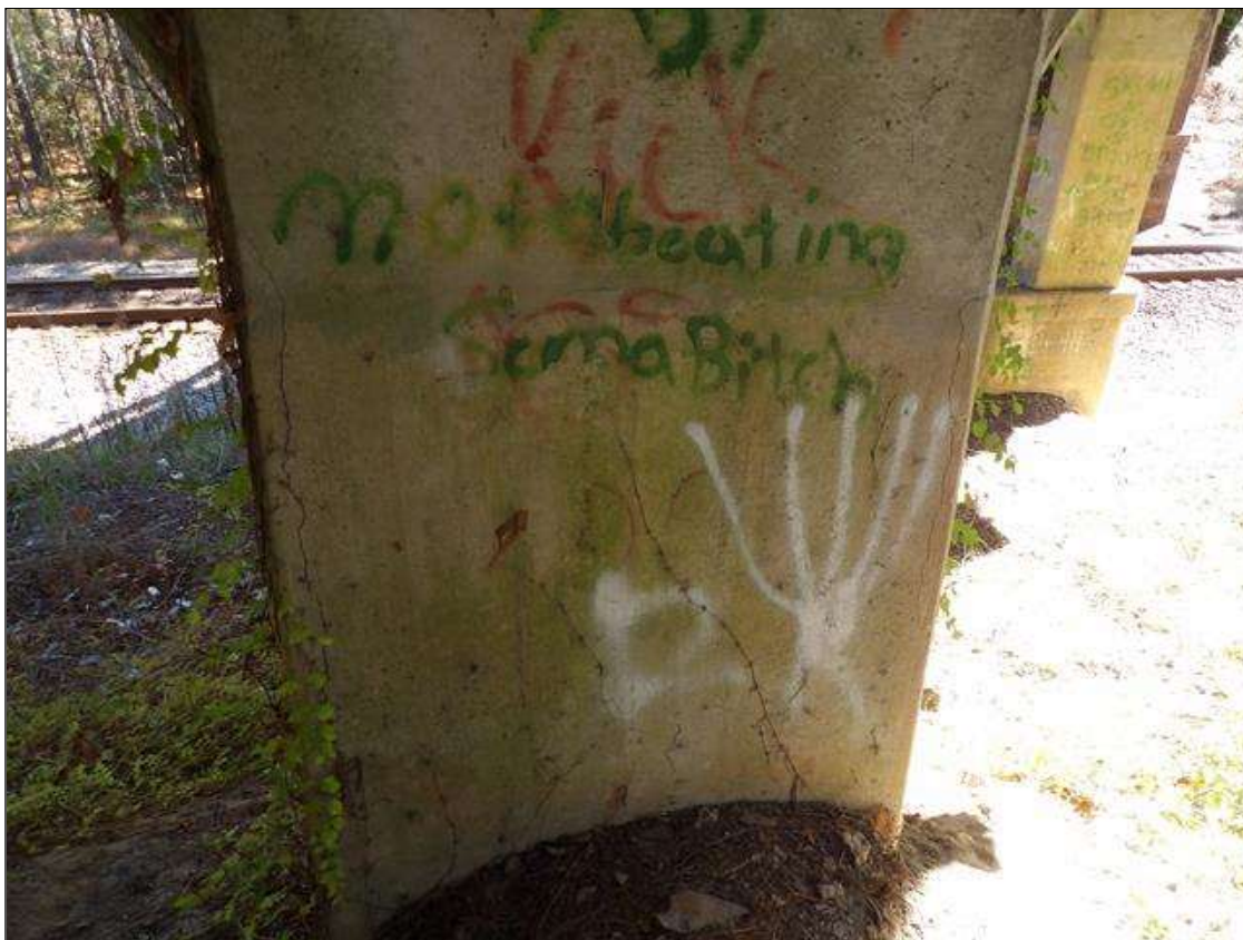
Bent 4 Pile 1: VERTICAL CRACK 5 FEET LONG UP TO 1/8 INCHES WIDE AT NORTHEAST AND NORTHWEST CORNERS
