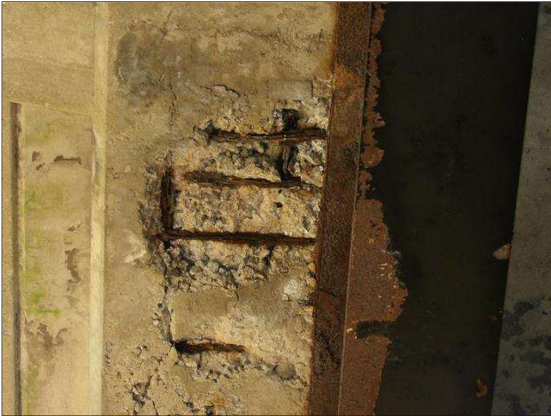
Span 3 Deck: PAR--3 FOOT LONG X 15 INCHES WIDE X 2 INCHES DEEP SPALL WITH EXPOSED REBAR IN UNDERSIDE OF LEFT OVERHANG NEAR MID SPAN. MULTIPLE EXPOSED BARS TRANSVERSE AND LONGITUDINAL HAVE SECTION LOSS WITH 50 PERCENT AREA REMAINING
