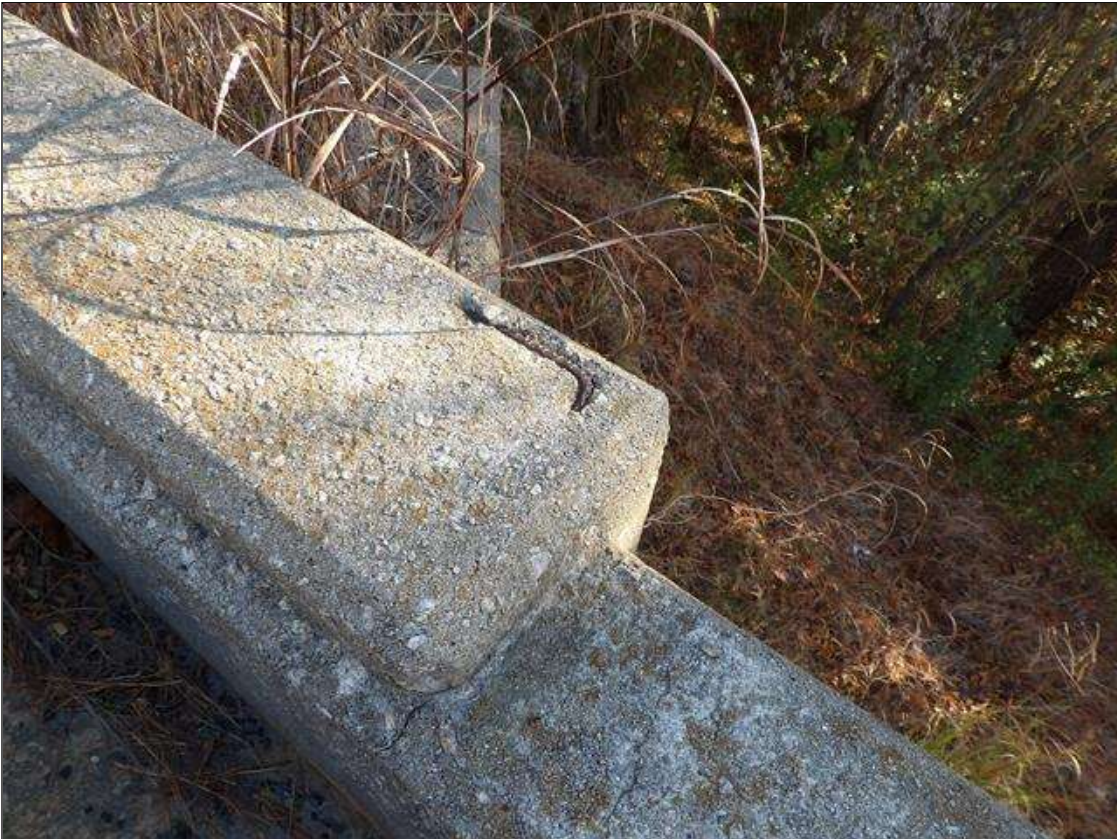
Span 5 Right Bridge Rail: FAR END ON THE TOP OF THE REINFORCED CONCRETE RAIL, EXPOSED REBAR [APPROXIMATELY 5 INCHES LONG X 1/2 INCHES WIDE] WITH NO MEASURABLE SECTION LOSS
