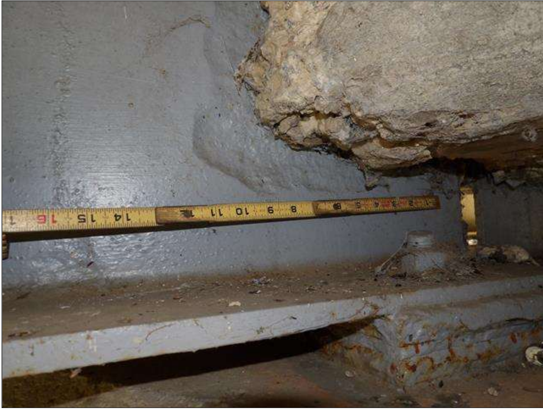
Span 5 Beam 2: PAR--1 FEET LONG X 2 INCHES WIDE AREA OF PREVIOUS CORROSION WITH 1/4 INCHES REMAINING SECTION IN WEB AROUND END DIAPHRAGM AT BENT 4 AREA HAS BEEN PAINTED OVER AND ARRESTED.
