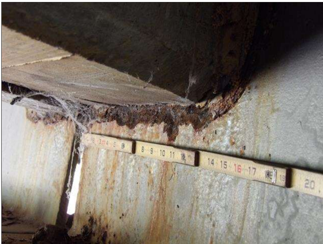
TYPICAL CORROSION UP TO 1/8 INCH LOSS X UP TO 2 FEET HIGH AT BEAM ENDS ADJACENT TO DIAPHRAGMS OVER PIERS WITH 7/16 INCH AVERAGE REMAINING. BEAM 3 SPAN 1 AT PIER 1 SHOWN
