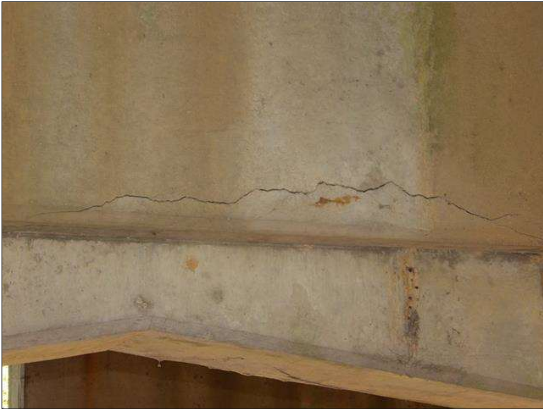
Bent 1 Cap 1: HORIZONTAL CRACK 3 FEET LONG UP TO 3/16 INCHES WIDE IN SOUTH FACE MID WAY BETWEEN COLUMNS 1 AND 2
