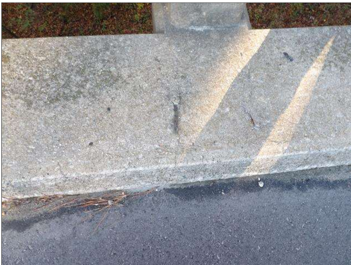
Span 4 Left Bridge Rail: 3 INCHES X 1 INCHES X 1/2 INCHES DEEP SPALL WITH EXPOSED REBAR NO LOSS IN TOP OF CURB AT 10 FEET FROM BENT 4
