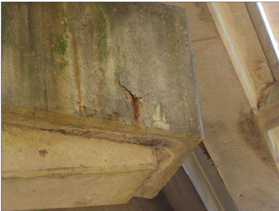
Bent 2 Cap 1: 8 INCHES DIAMETER DELAMINATION AND 6 INCHES DIAMETER X 1/2 INCHES DEEP SPALL WITH EXPOSED REBAR NO LOSS IN NORTH FACE UNDER BEAM 1
