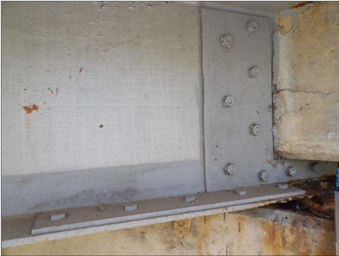
BOLTED PLATE REPAIR TO BOTTOM FLANGE WEST AND BOTH FACES OF WEB AT BENT 4 SPAN 5 BEAM 1
