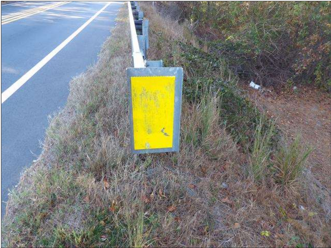
GUARDRAIL TERMINAL END NORTHWEST CORNER ALL OTHERS SIMILAR
