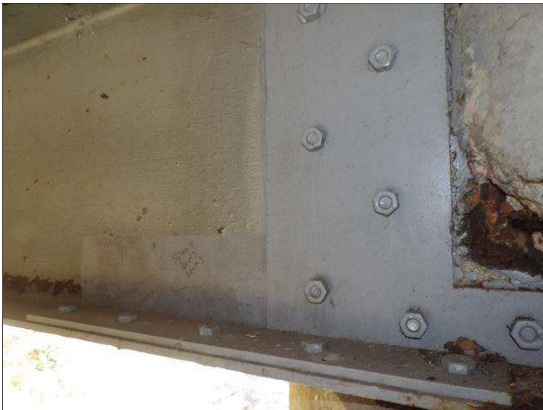
BOLTED PLATE REPAIR 24 INCH X 24 INCH TO WEB BOTH SIDES AND 24 INCH BOTTOM FLANGE WEST SIDE BEAM 5 SPAN 4 AT BENT 3
