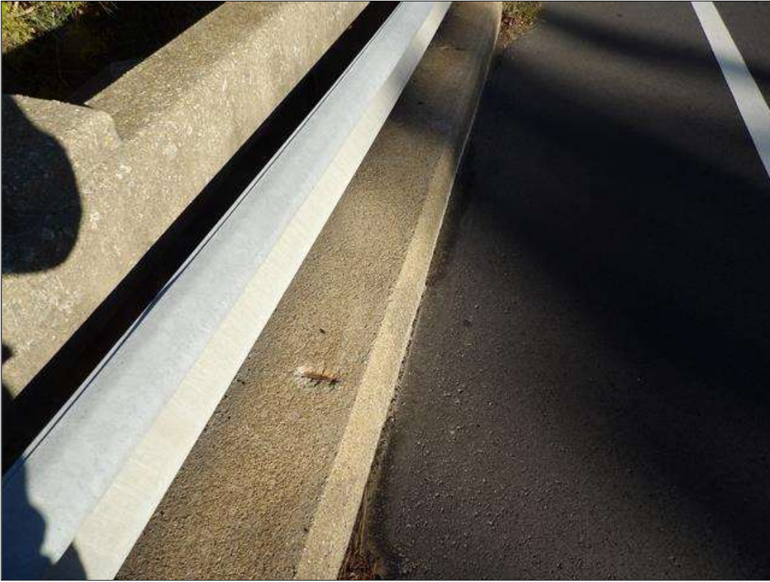
Span 5 Left Bridge Rail: TWO SPALLS WITH EXPOSED REBAR NO LOSS 3 INCHES X 1 INCHES X 1/2 INCHES DEEP IN TOP OF CURB AT 12 FEET AND 6 FEET FROM END BENT 2
