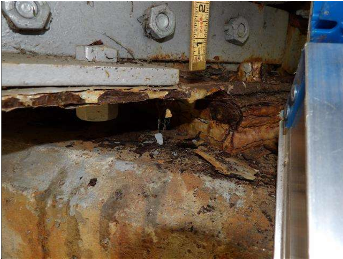
Span 5 Beam 1: PAR--1/4 INCH SECTION LOSS WITH 3/8 INCHES AVERAGE REMAINING FULL WIDTH OF BOTTOM FLANGE. BEAM END HAS BEEN PAINTED WITH ACTIVE SURFACE CORROSION PRESENT. BOLTED REPAIR REPAIR PLATE ADDED AND DOES NOT EXTEND UNDER DEFECT AT PIER 4.
