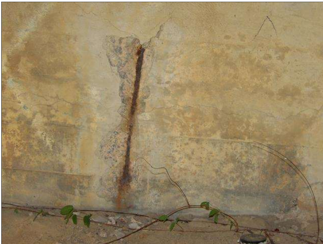
End Bent 1 Cap 1: 8 INCHES X 2 FEET X 3/4 INCHES DEEP SPALL WITH EXPOSED REBAR NO LOSS UNDER BAY 4
