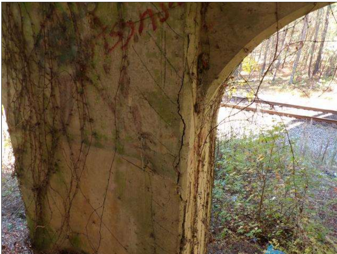
Bent 4 Pile 2: 6 FOOT X 9 INCH AREA OF DELAMINATION AT NORTHWEST CORNER
