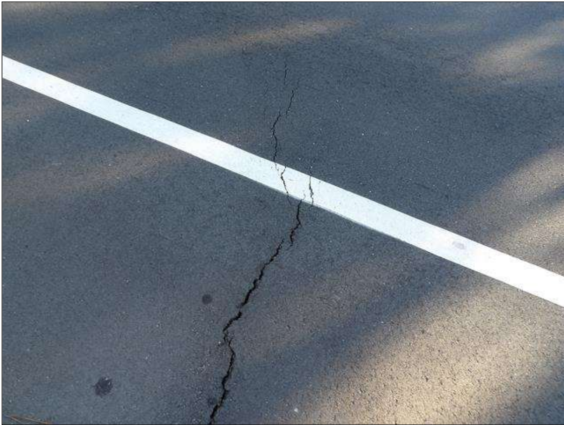
Span 4 Wearing Surface: FULL WIDTH TRANSVERSE/MP CRACKING UP TO 1/4 INCHES WIDE OVER BENT 4,
