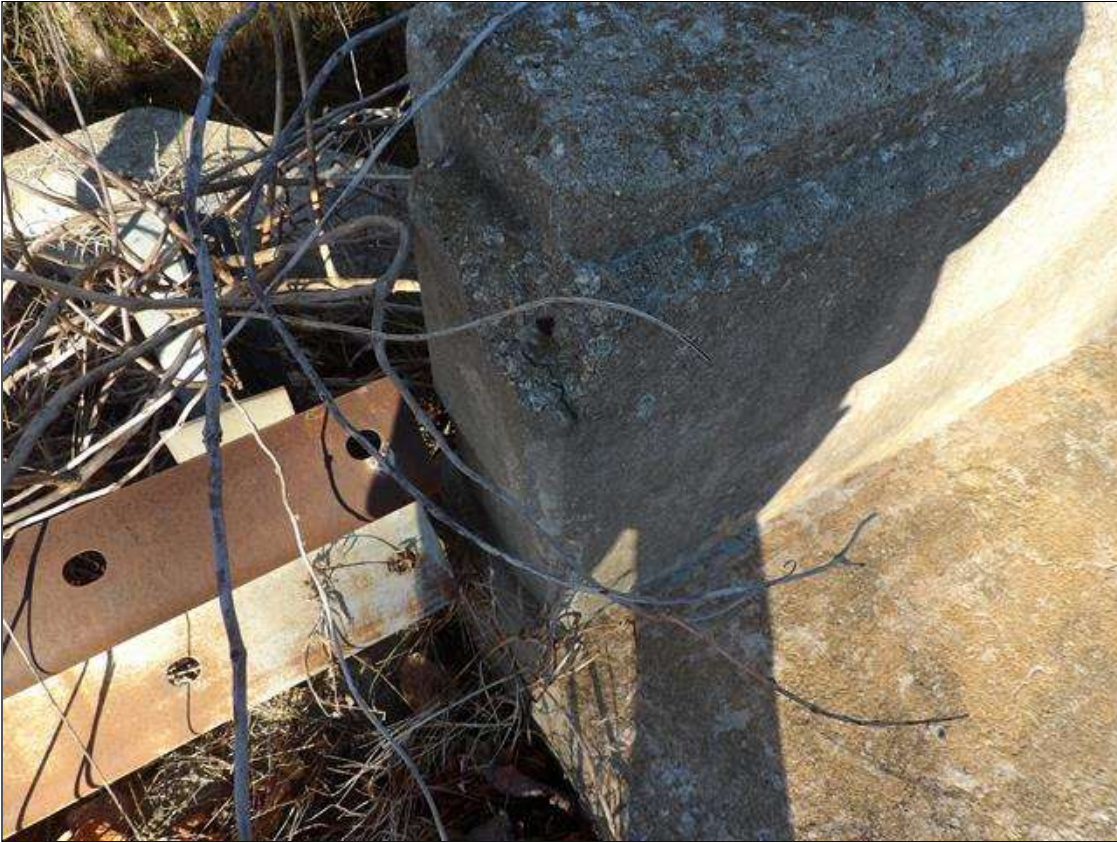
Span 1 Left Bridge Rail: 4 INCHES DIAMETER X 1 INCHES DEEP SPALL WITH EXPOSED REBAR NO LOSS AT END POST AT SOUTHWEST CORNER
