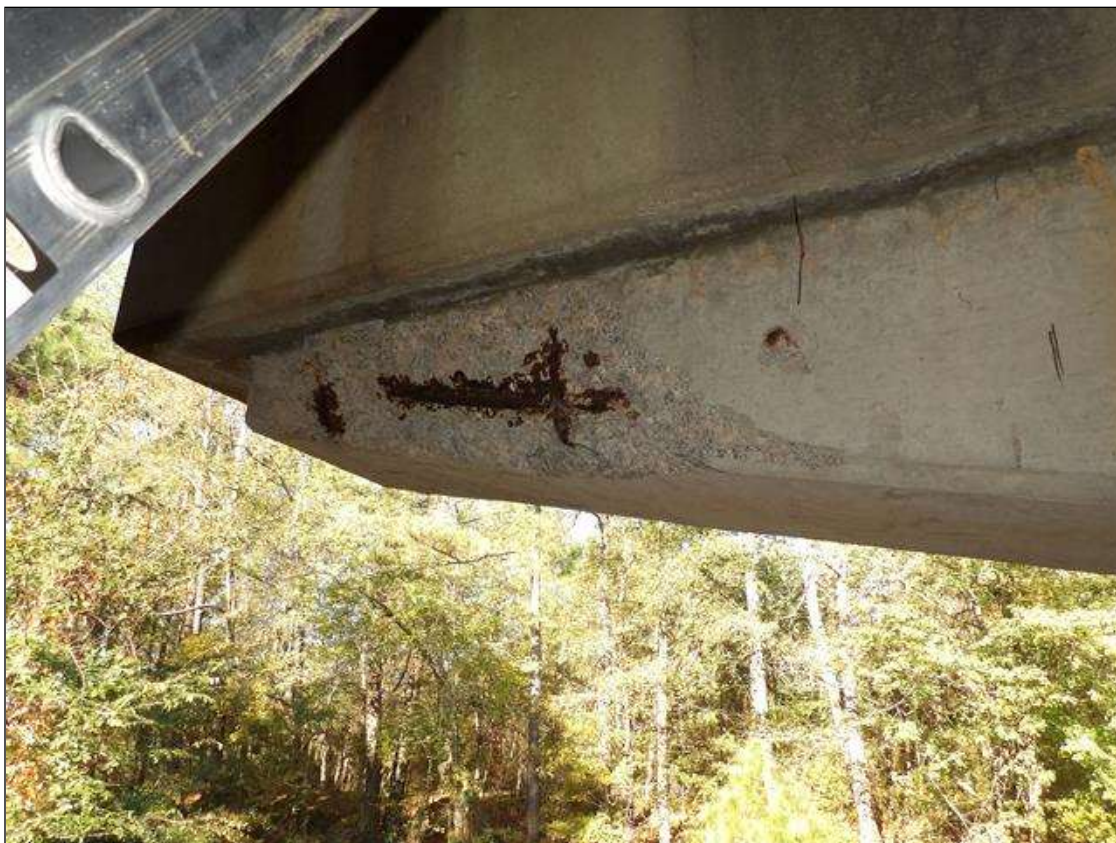
Bent 1 Cap 1: SOUTH FACE AT THE LEFT END, LOWER 10 INCHES, SPALLING WITH EXPOSED REBAR NO MEASURABLE SECTION LOSS [APPROXIMATLY 40 INCHES LONG X UP TO 2.5 INCHES DEEP]
