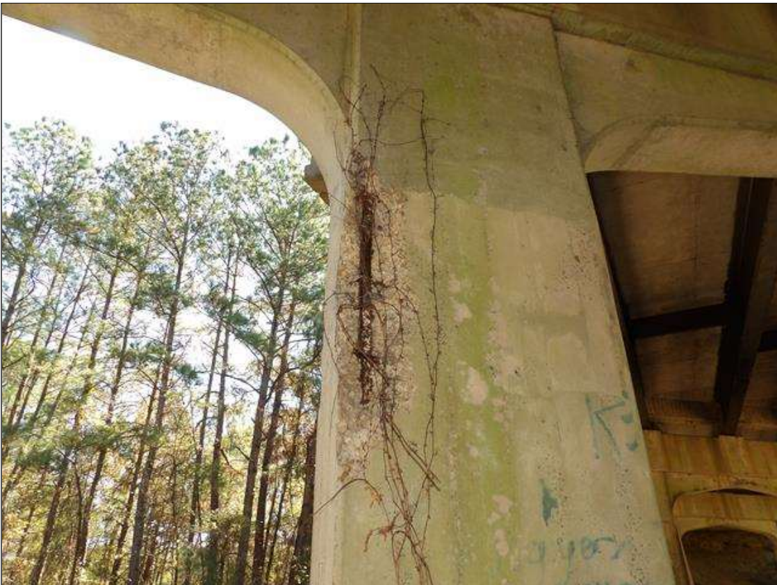
Bent 3 Pile 2: PAR--SPALL WITH EXPOSED REBAR AND BROKEN HORIZONTAL TIE 3 FOOT X 1 FOOT X 4 INCHES DEEP IN NORTHEAST CORNER MID HEIGHT WITH SECTION LOSS
