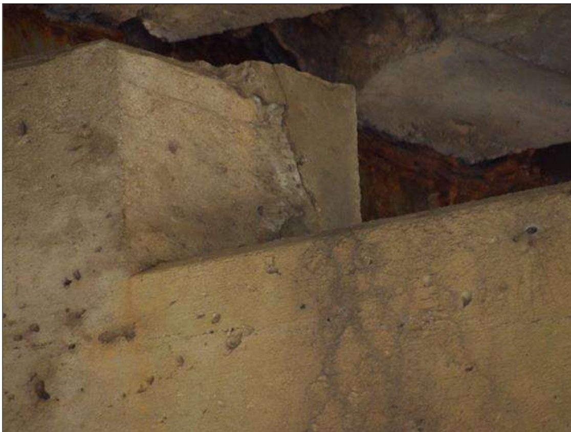
Bent 2 Cap 1: 8 INCH X 6 INCH SOUND PATCH EAST FACE OF PEDESTAL UNDER BEAM 2, PEDESTAL UNDER BEAM 3 SIMILAR
