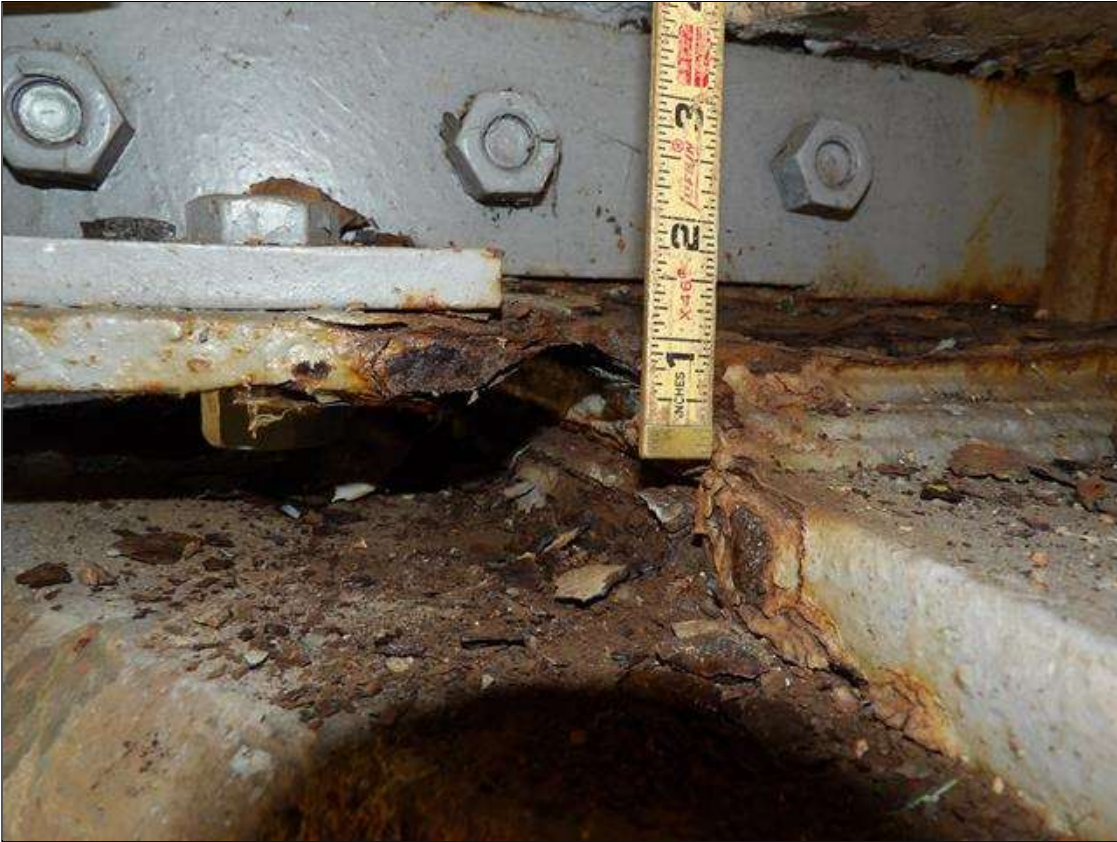
Span 4 Beam 5: PAR--SECTION LOSS UP TO 3/8 INCHES WITH 3/8 INCHES AVERAGE REMAINING FULL WIDTH OF BOTTOM FLANGE 1 FEET LONG ON BEAM END OVER PIER 3. BEAM END HAS BEEN CLEANED AND PAINTED WITH ACTIVE SURFACE CORROSION. PLATE REPAIR ADDED BUT DOES NOT EXTEND OUT TO DEFECT.
