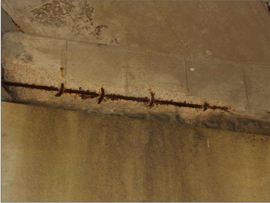
TYPICAL DIAPHRAGM SPALL UP TO 4 FOOT LONG X 1 FOOT HIGH X 4 INCHES DEEP WITH EXPOSED REBAR NO LOSS OVER PIERS, SPAN 2 BAY 4 OVER PIER 1 SHOWN
