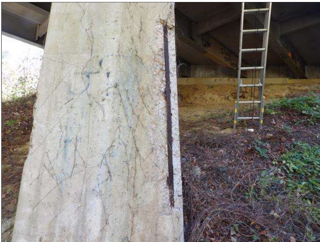
Bent 1 Pile 1: 6 FOOT X 9 INCHES X 2 INCHES DEEP SPALL WITH EXPOSED RUSTED REBAR NO SECTION LOSS AT NORTHWEST CORNER
