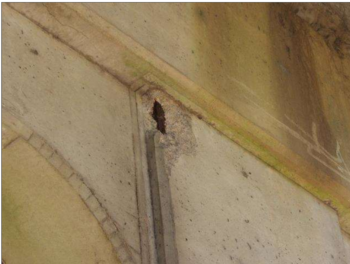
Bent 2 Pile 2: SPALL 10 INCH X 9 INCH X 2 INCH DEEP WITH EXPOSED REBAR NO LOSS AT TOP SOUTHWEST CORNER
