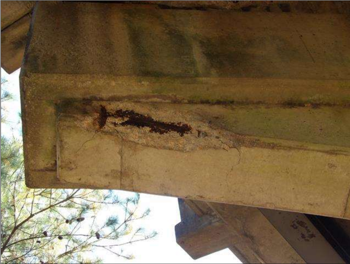
Bent 2 Cap 1: 3 FEET X 1 FEET X 6 INCHES DELAMINATION WITH A SPALL 2 FOOT X 9 INCH X 3 INCH DEEP WITH EXPOSED REBAR NO LOSS IN UNDERSIDE UNDER BEAM 5 IN FLUTED PORTION
