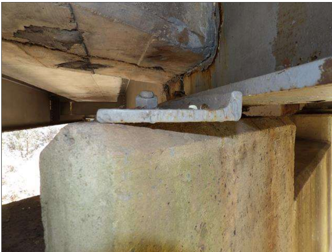
2 FOOT LONG X 6 INCH WIDE BRACE PLATE ON TOP OF PEDESTAL AT PIER 3 RIGHT SIDE OF NEAR BEARING BEAM 4 SPAN 4
