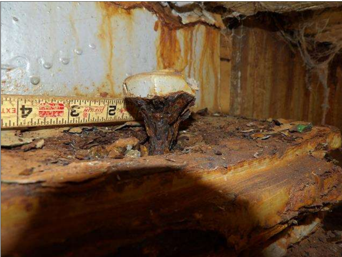
Span 4 Near Bearing 2: PAR--UP TO 50 PERCENT SECTION LOSS ON LEFT ANCHOR BOLT
