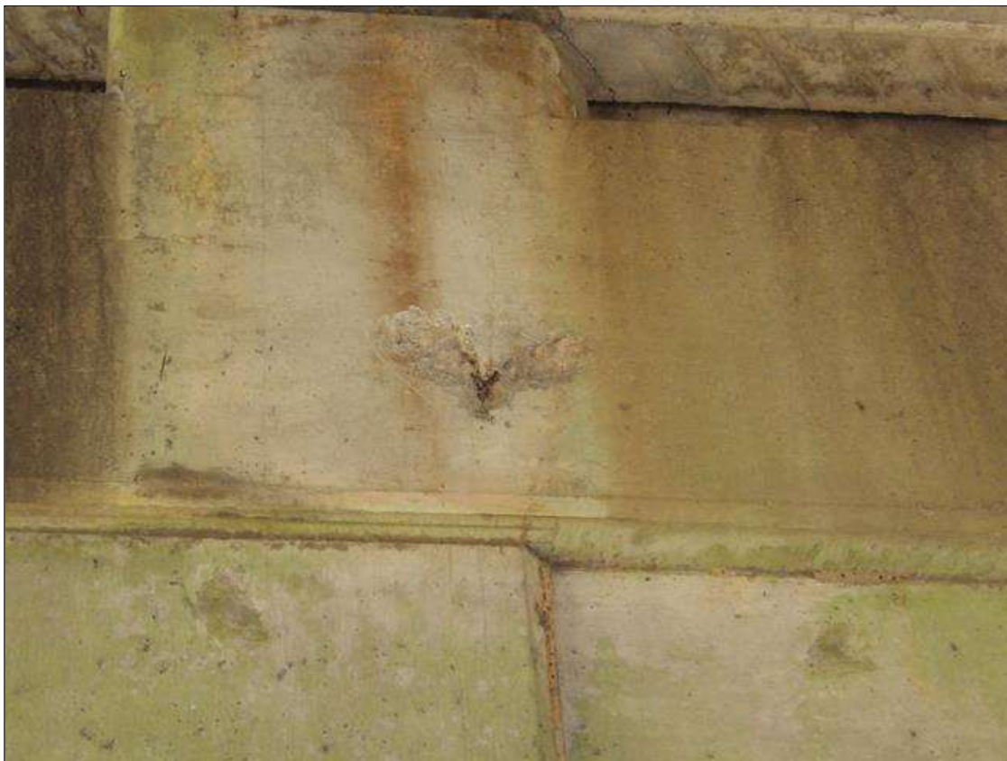
Bent 3 Cap 1: SPALL WITH EXPOSED REBAR NO LOSS 1 FEET X 9 INCHES X 1 INCHES DEEP IN NORTH FACE UNDER BEAM 4
