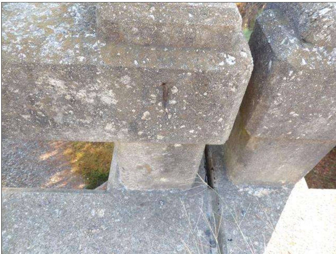
Span 3 Right Bridge Rail: 3 INCHES X 1 INCHES X 1/2 INCHES DEEP SPALL WITH EXPOSED REBAR NO LOSS IN FACE OF RAIL POST AT BENT 2
