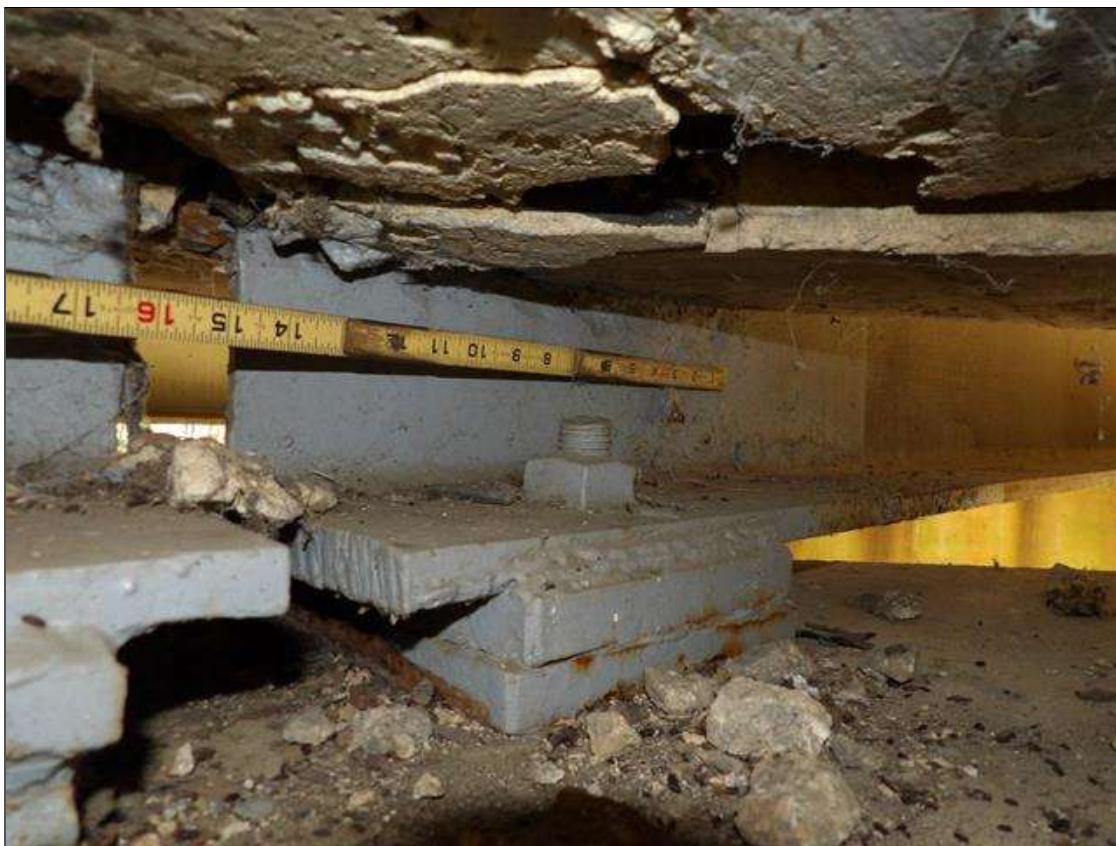
Span 4 Beam 2: PAR--BEAM END AT BENT 4 AT THE INTERFACE WITH THE REINFORCED CONCRETE DIAPHRAGM, THERE IS A BAND OF CORROSION UP TO 1 INCHES WIDE WITH SECTION LOSS [AVERAGE 3/8 INCHES REMAINS] FOR APPROXIMATELY 1 FEET LONG X UP TO THE FULL HEIGHT OF THE DIAPHRAGM.
