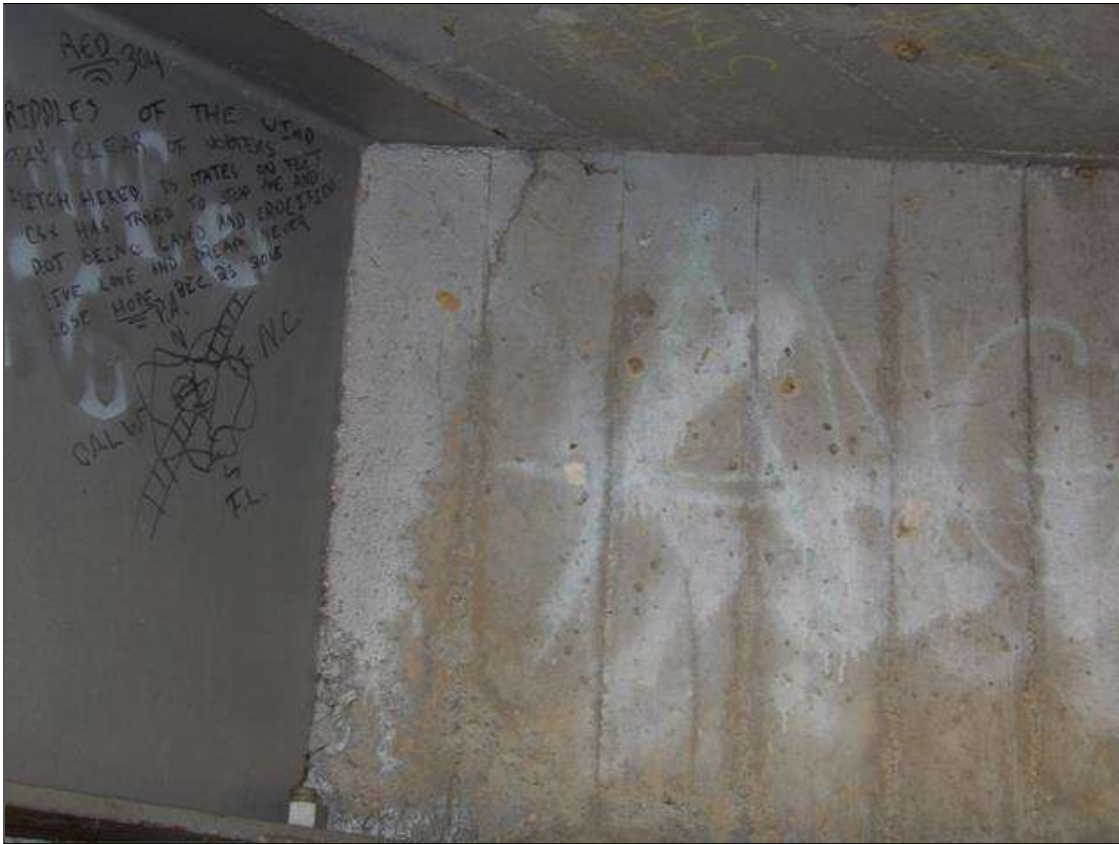
End Bent 1 Abutment: 1 FEET LONG VERTICAL HAIRLINE TO 1/32 INCHES CRACK BAY 3
