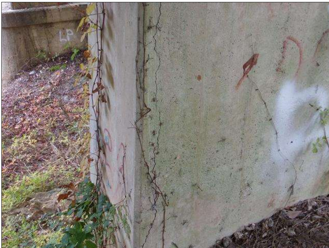
Bent 4 Pile 1: VERTICAL CRACK 5 FT LONG UP TO 1/8" WIDE AT NORTHEAST CORNER
