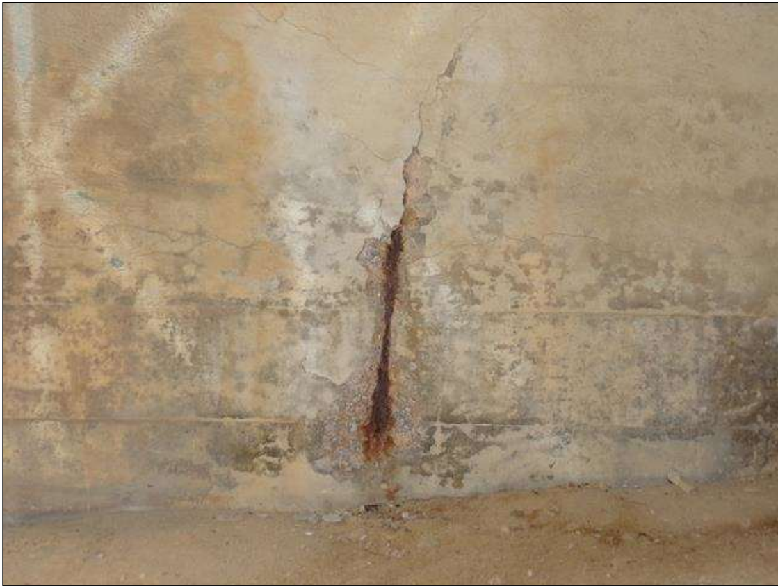
End Bent 1 Cap 1: 8" X 2 FT X 1/2" DEEP SPALL WITH EXPOSED REBAR UNDER BAY 4
