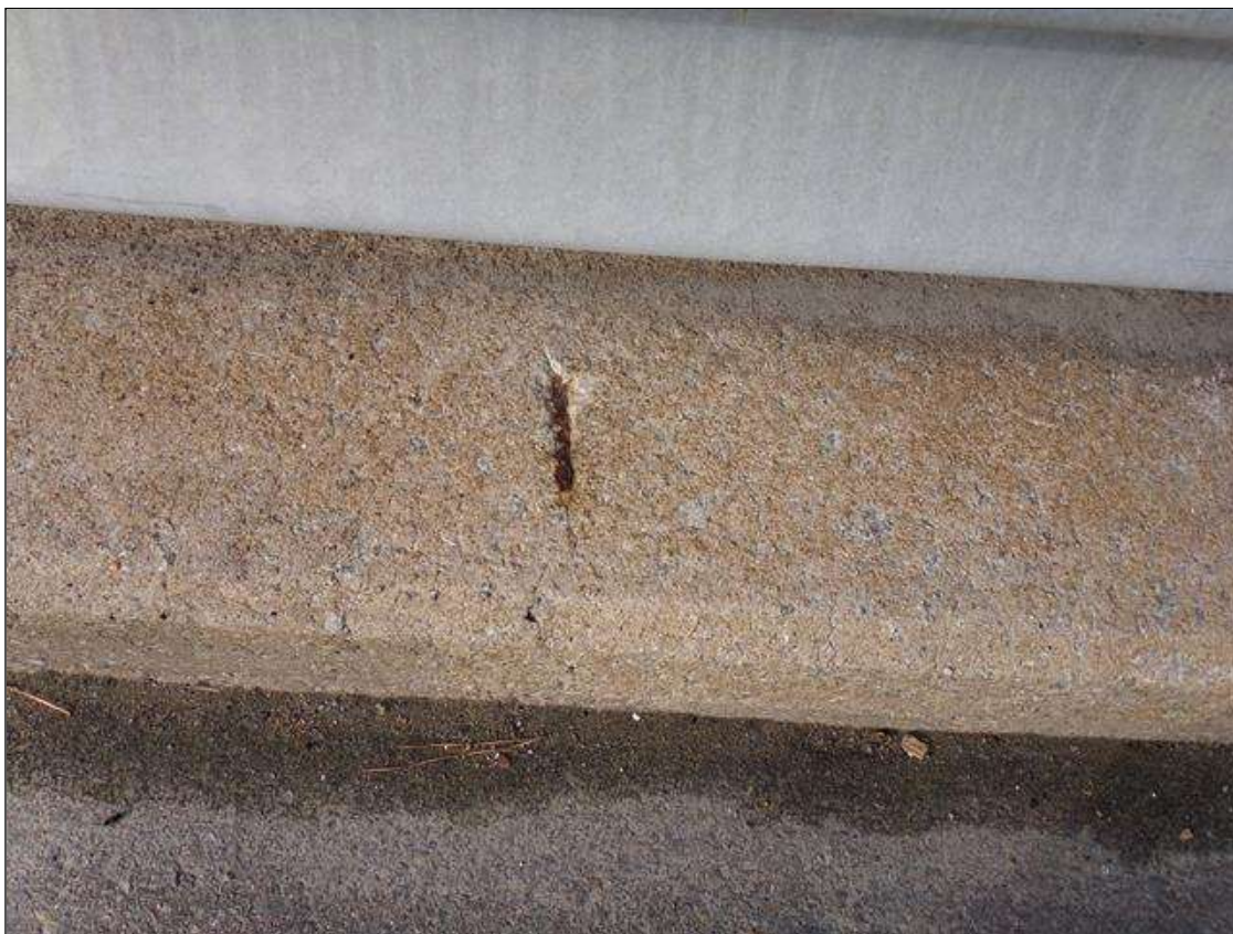
Typical small surface spall with exposed rebar in top of curb, span 5 left rail shown
