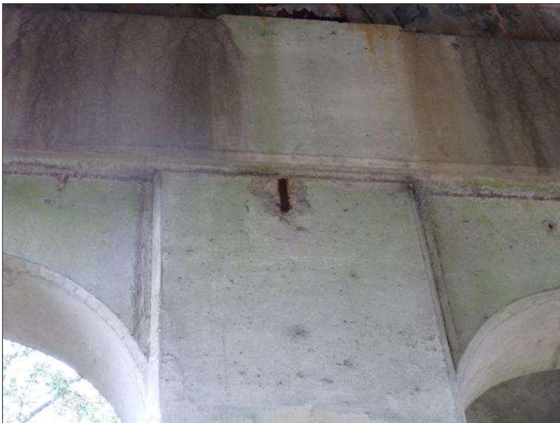
Bent 3 Pile 1: 9" X 6" X 1/2" DEEP SPALL WITH EXPOSED REBAR NO LOSS IN SOUTH FACE BELOW CAP
