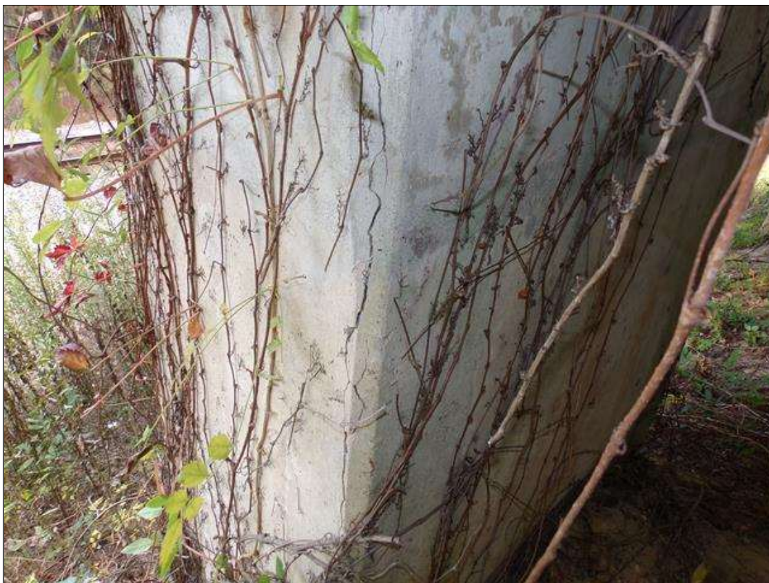
Bent 4 Pile 2: 6 FT X 9" AREA OF DELAMINATION WITH CRACKING UP TO 1/8" WIDE AT NORTHEAST CORNER
