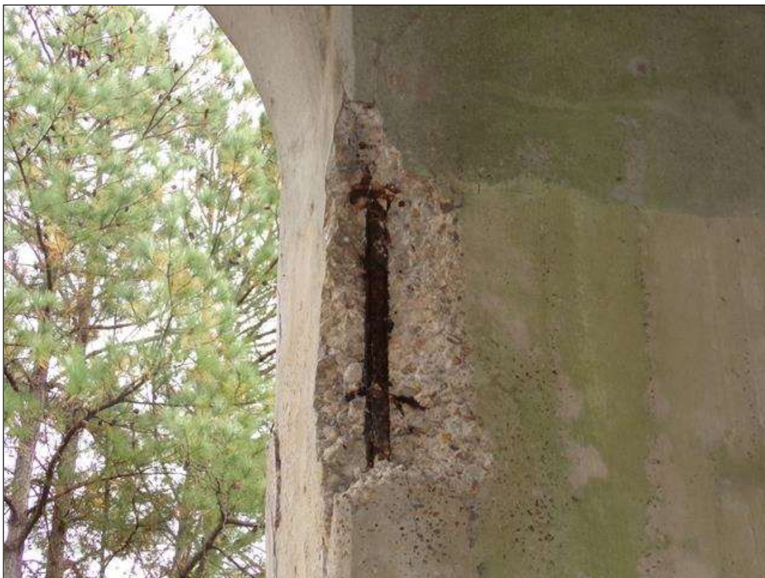
Bent 3 Pile 2: PAR--SPALL WITH EXPOSED REBAR AND BROKEN HORIZONTAL TIE 3 FT X 1 FT X 4" DEEP IN NORTHEAST CORNER MID HEIGHT WITH SECTION LOSS
