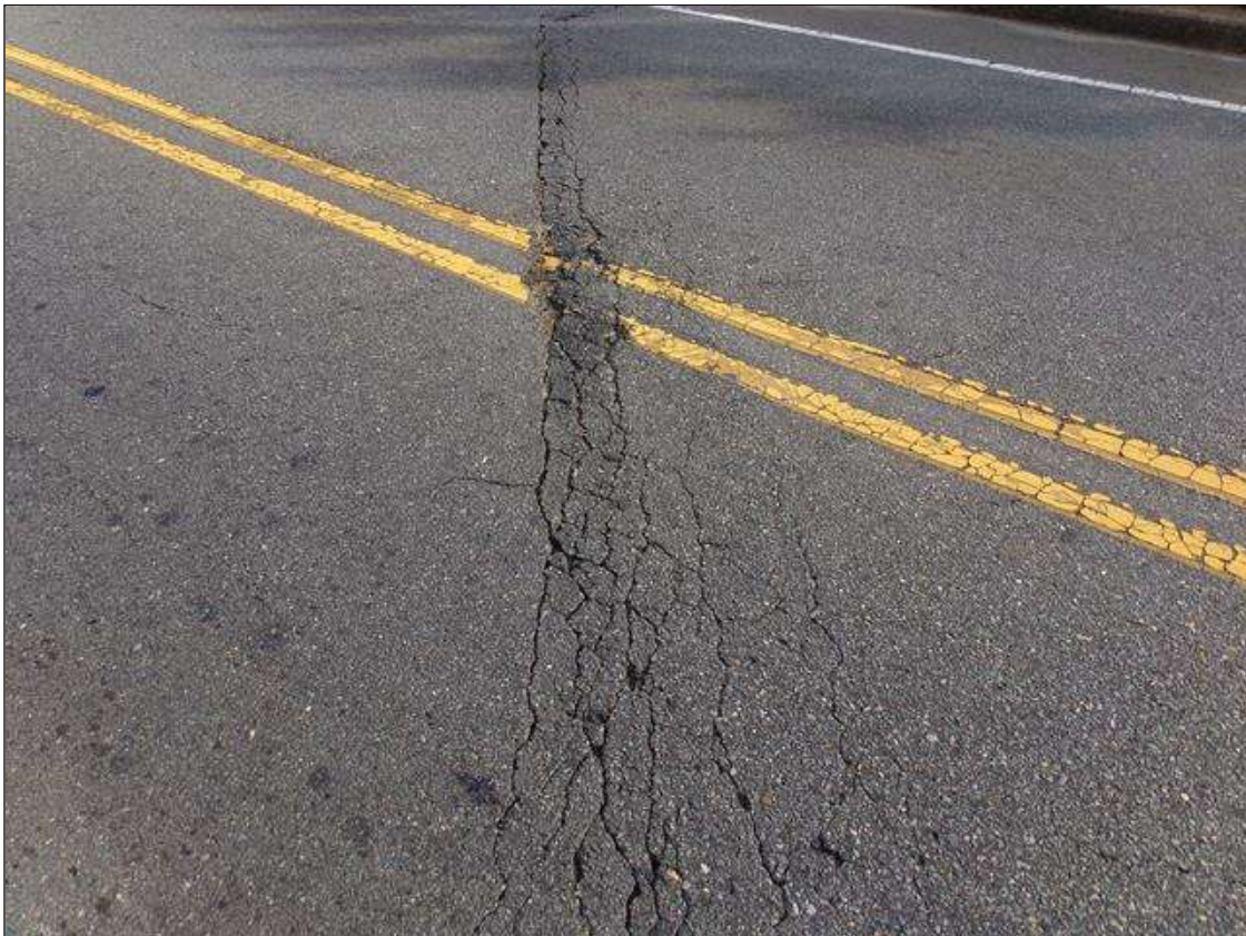
Span 3 Wearing Surface: FULL WIDTH TRANSVERSE/MAP CRACK UP TO 2" WIDE WITH ASPHALT DETERIORATION WITH UP TO 3/4" DEEP POT HOLES UP TO 1' LONG X 2" WIDE OVER BENT 3
