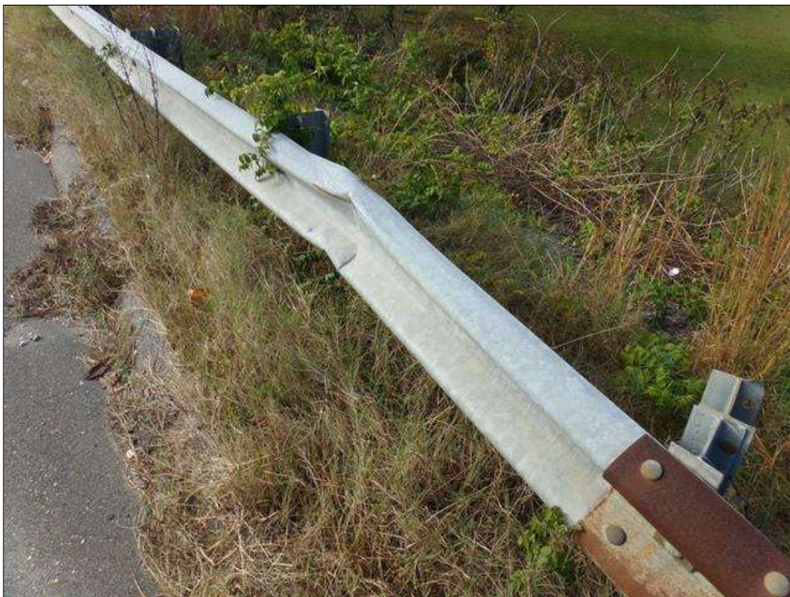
Guardrail impact damage to southwest rail midway 10' long
