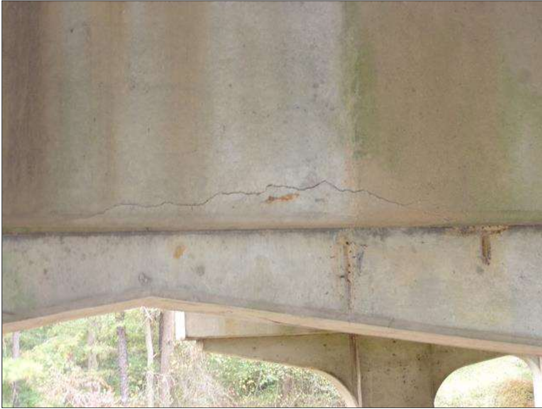
Bent 1 Cap 1: HORIZONTAL CRACK 3 FT LONG UP TO 1/8" WIDE IN SOUTH FACE MID WAY BETWEEN COLUMNS 1 AND 2
