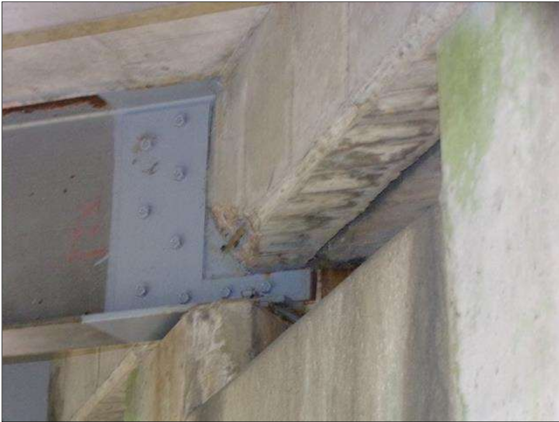
BOLTED PLATE REPAIR TO WEB ON BEAM 3 SPAN 4 24" X 24" AT BENT 3 END BOTH FACES
