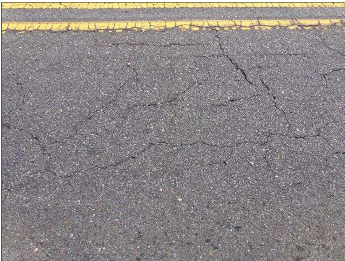
Span 1 Wearing Surface: Full length longitudinal/map cracking up to 1/4" wide in travel lanes
