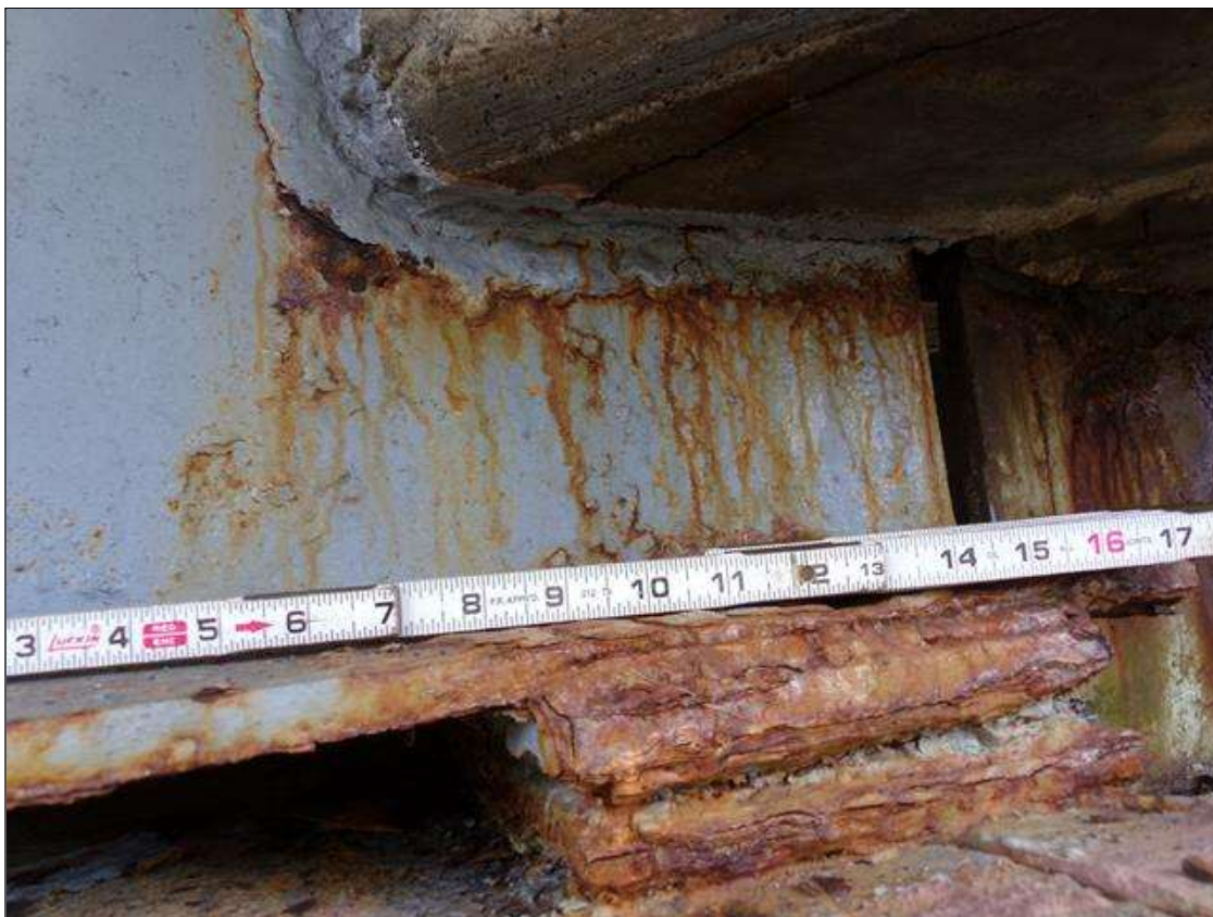
Span 2 Beam 5: 1 FT. OF PREVIOUS CORROSION WITH 1/2" X FULL WIDTH REMAINING SECTION IN BOTTOM FLANGE AND 7/16" REMAINING SECTION IN WEB AROUND END DIAPHRAGM AT BENT 2 HAS BEEN PAINTED WITH ACTIVE SURFACE CORROSION
