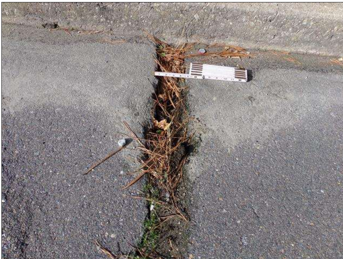
Span 4 Wearing Surface: 3' Long x 6" wide x 2 1/2" deep pothole at left shoulder at pier 3
