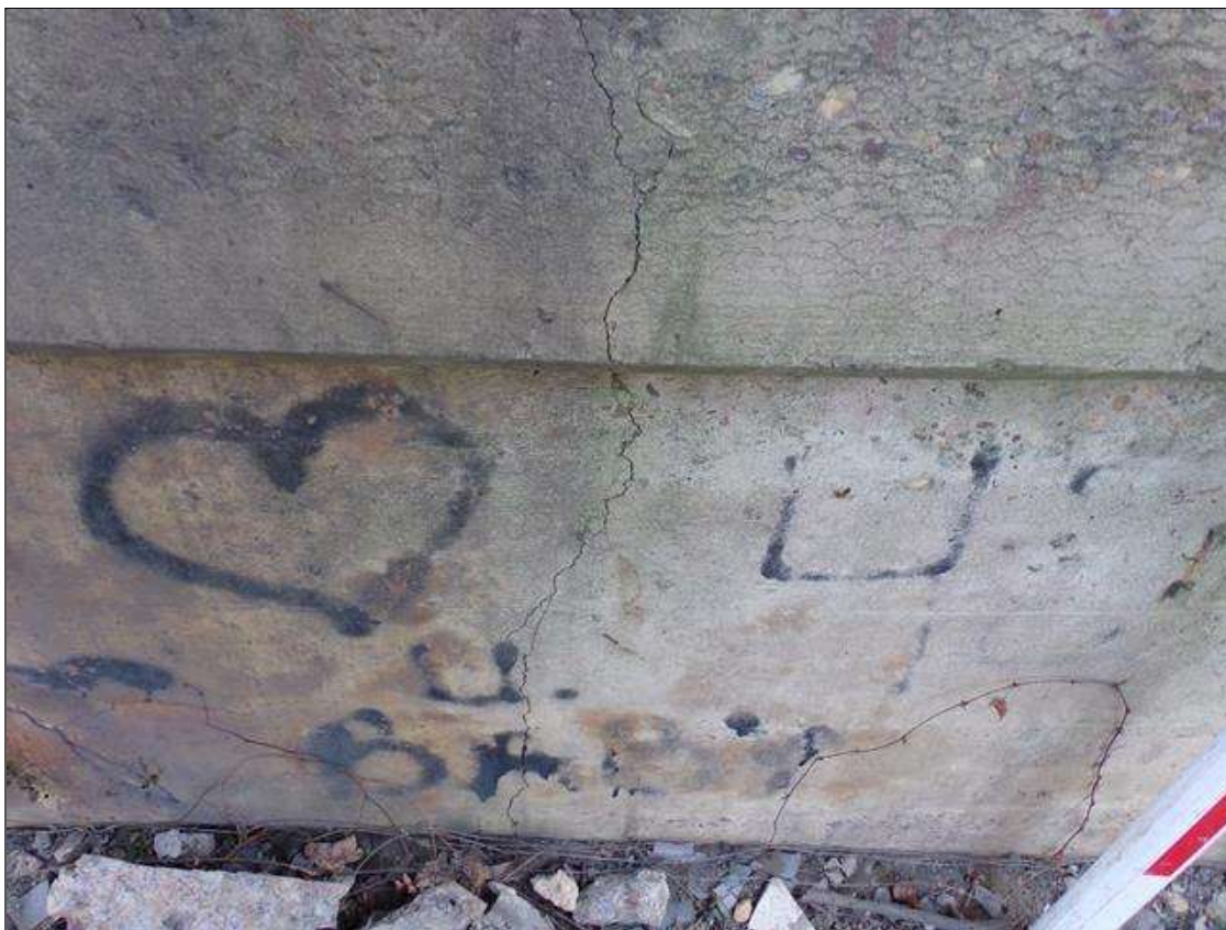
Bent 3 Pile 1: VERTICAL THRU CRACK 7 FT LONG X 1/8" WIDE IN MIDDLE OF CRASHWALL BOTH FACES
