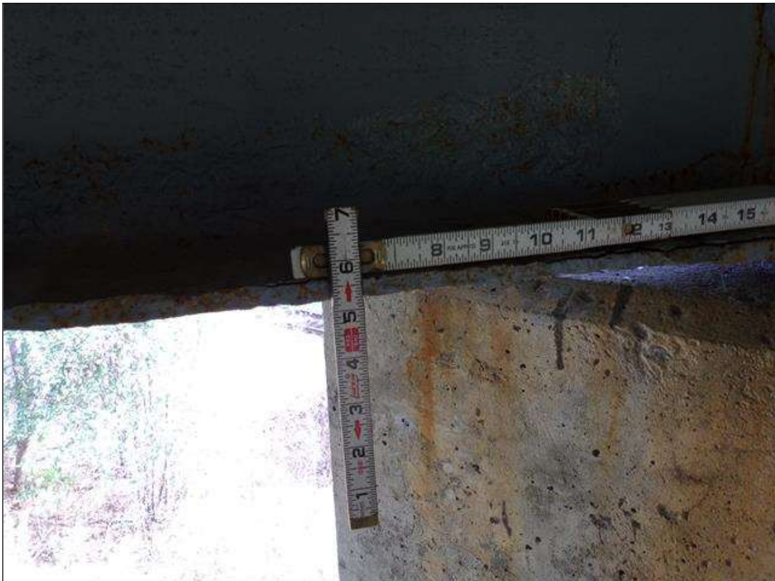
Span 5 Beam 5: PAR--1/4" section loss with 3/8" average remaining full width of bottom flange 4' long. Beam end has been painted with rust staining present at pier 4.
