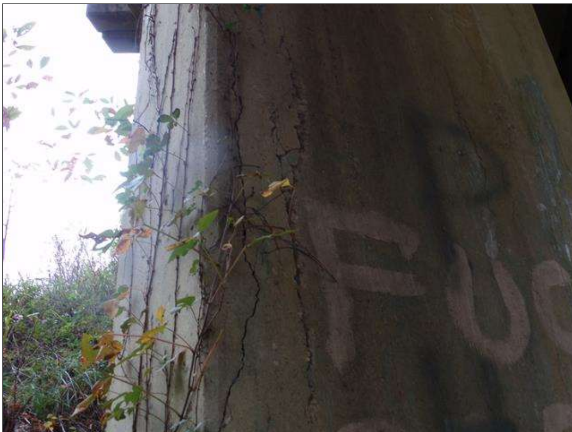
Bent 1 Pile 2: 4 FT X 1 FT X 1/2" DEEP SPALL AND DELAMINATION WITH CRACKS UP TO 1/8" WIDE IN NORTH FACE
