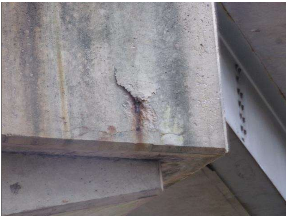
Bent 2 Cap 1: 8" DIAMETER DELAMINATION AND 6" DIAMETER X 1/2" DEEP SPALL WITH EXPOSED REBAR NO LOSS IN NORTH FACE UNDER BEAM 1
