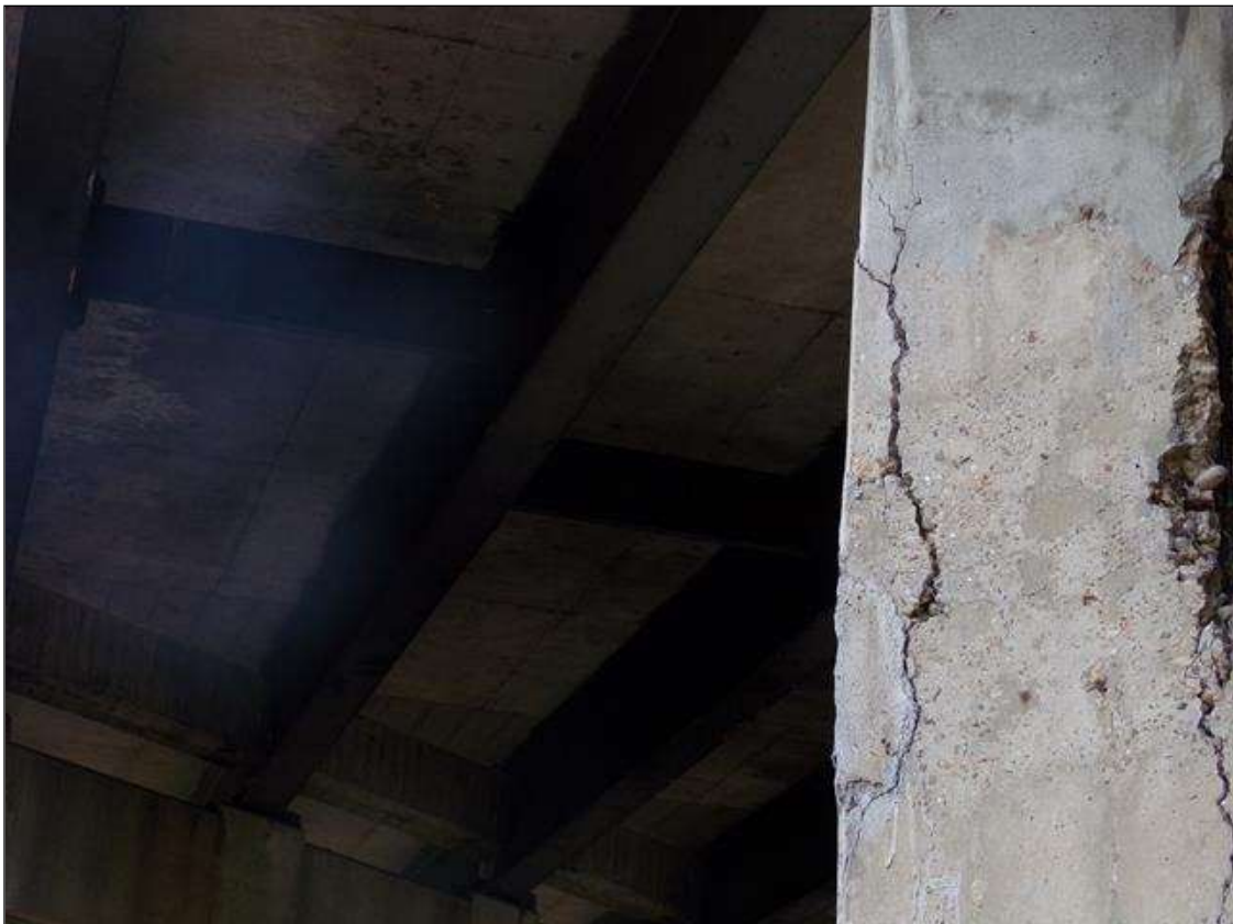
Bent 3 Pile 2: 4 FT X 2 FT AREA OF DELAMINATION WITH CRACKING UP TO 1/2" WIDE AT SOUTHEAST CORNER
