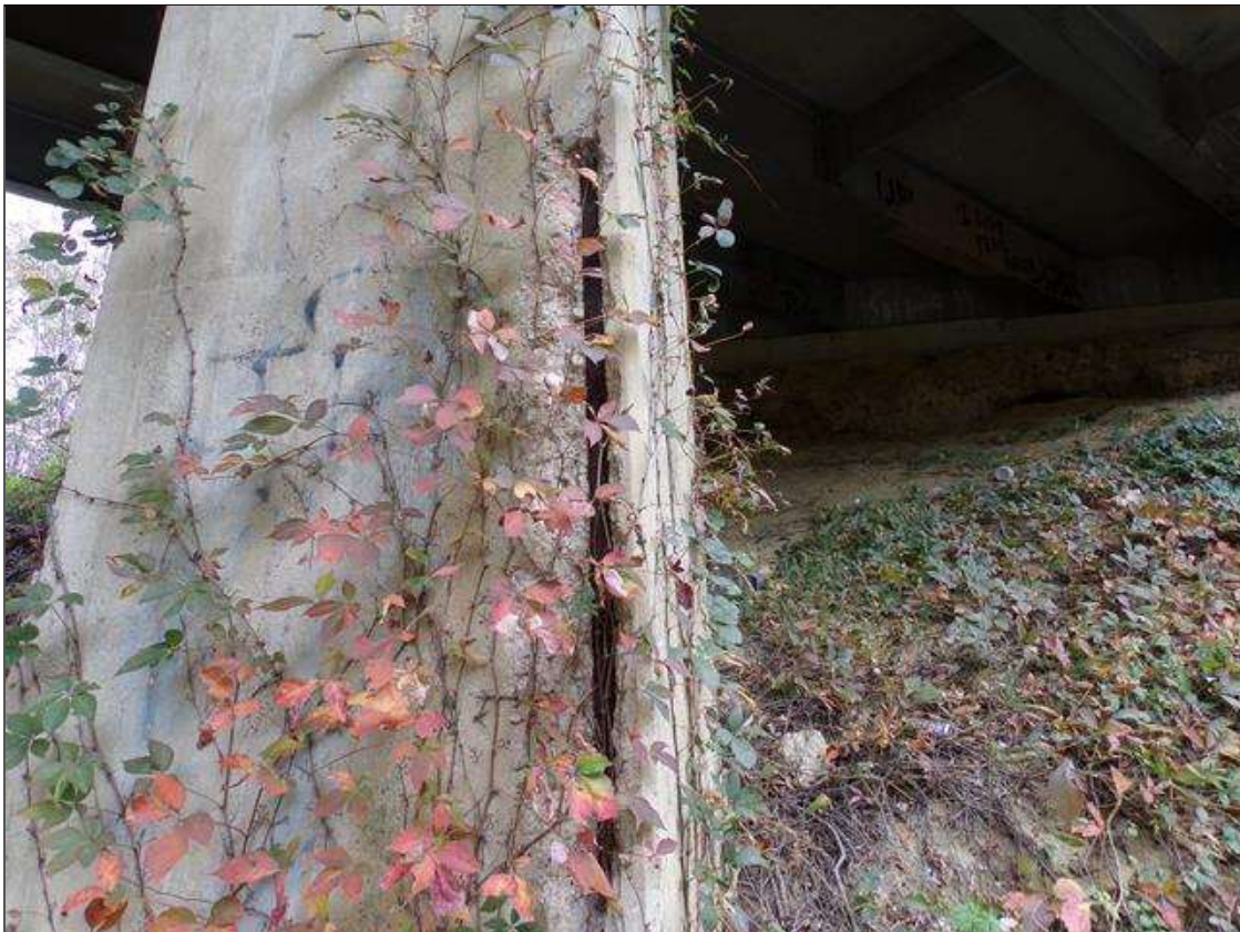
Bent 1 Pile 1: 6 FT X 9" FT X 2" DEEP SPALL WITH EXPOSED RUSTED REBAR NO SECTION LOSS AT NORTHWEST CORNER
