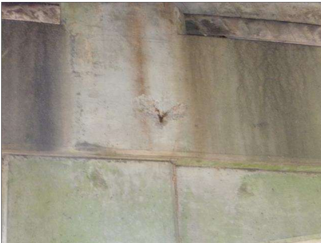
Bent 3 Cap 1: SPALL WITH EXPOSED REBAR 1 FT X 9" X 1" DEEP IN NORTH FACE UNDER BEAM 4
