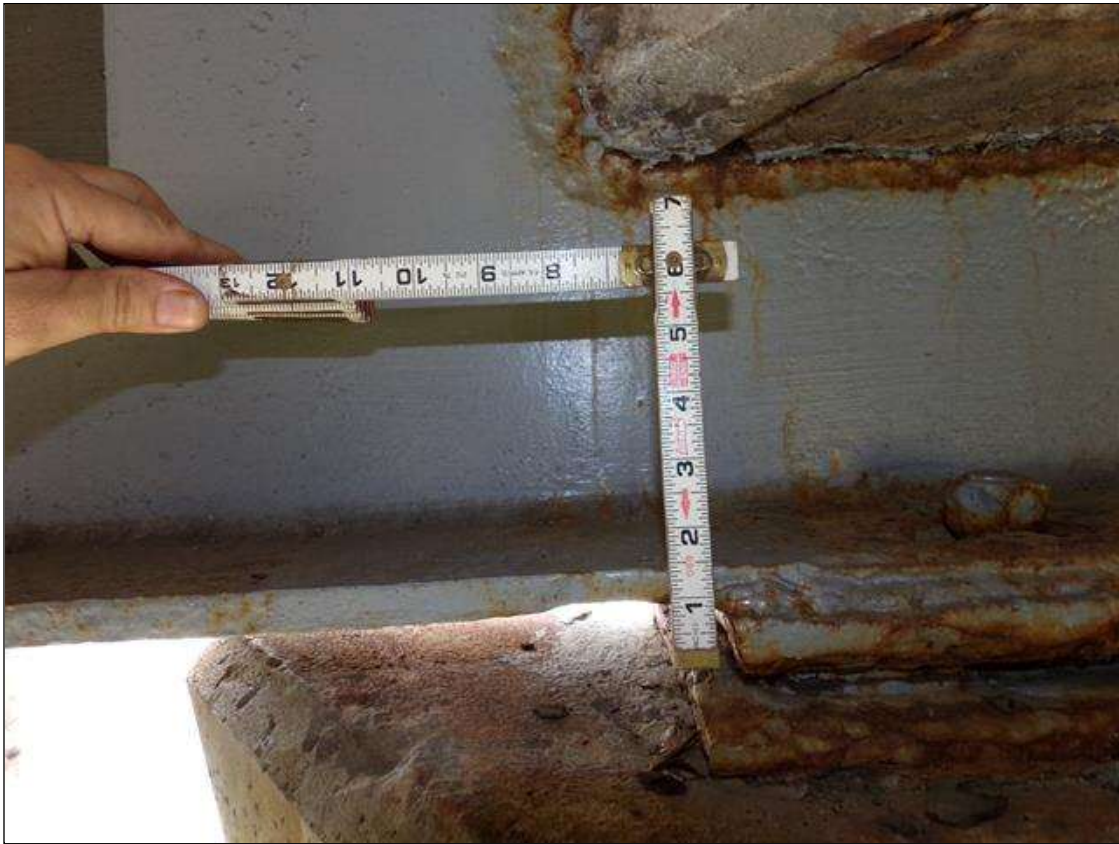
Span 2 Beam 1: 1 FT. OF PREVIOUS CORROSION WITH 1/2" REMAINING SECTION IN BOTTOM FLANGE AND 7/16" REMAINING SECTION IN WEB AROUND END DIAPHRAGM AT BENT 2 HAS BEEN PAINTED OVER AND ARRESTED.
