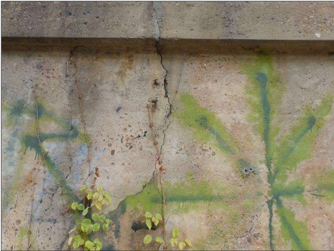
Bent 3 Pile 1: VERTICAL THRU CRACK 7 FT LONG X 1/4" WIDE IN MIDDLE OF CRASHWALL BOTH FACES
