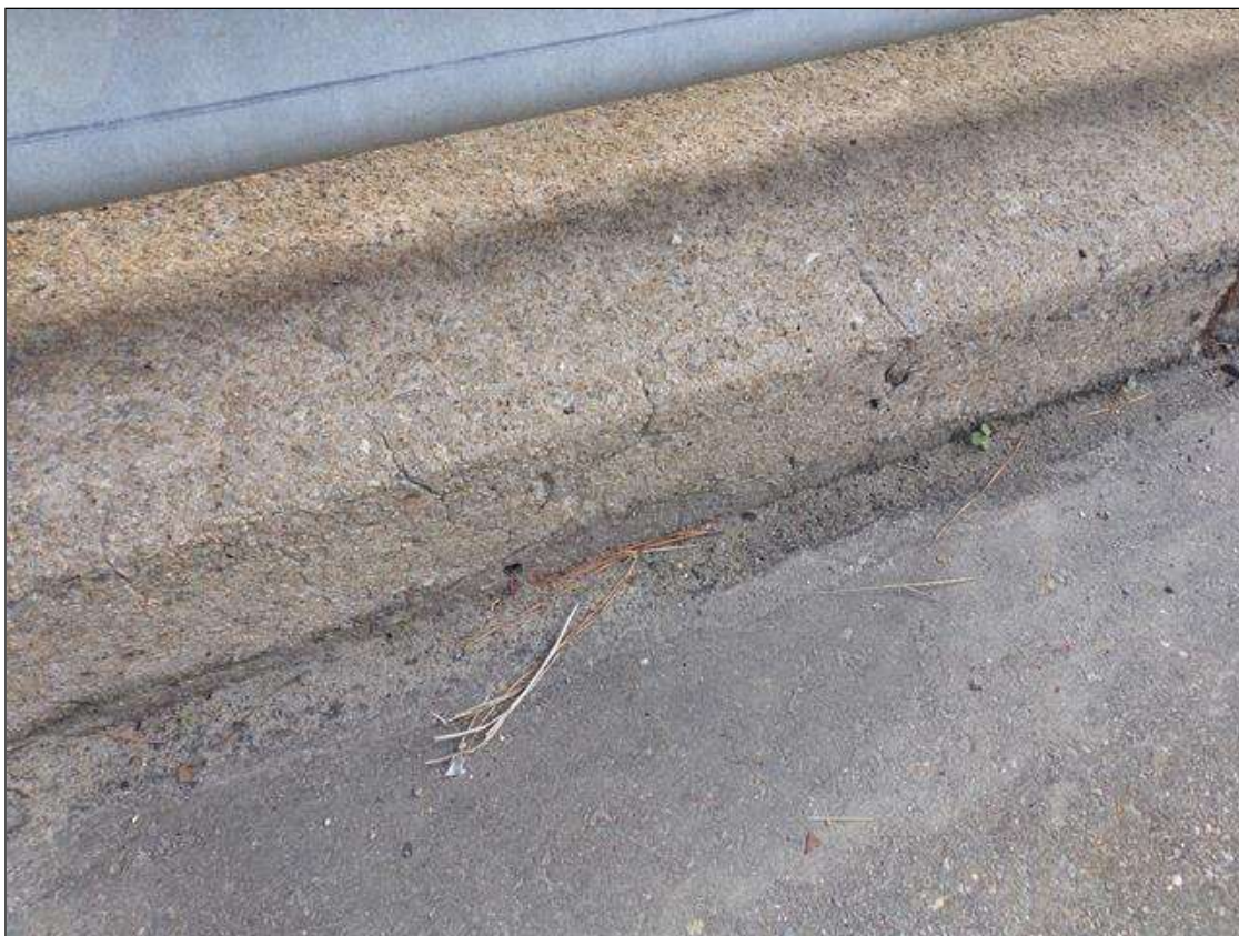
Typical hairline to 1/16" wide transverse/map cracking in curb portion of rail, right rail span 5 shown
