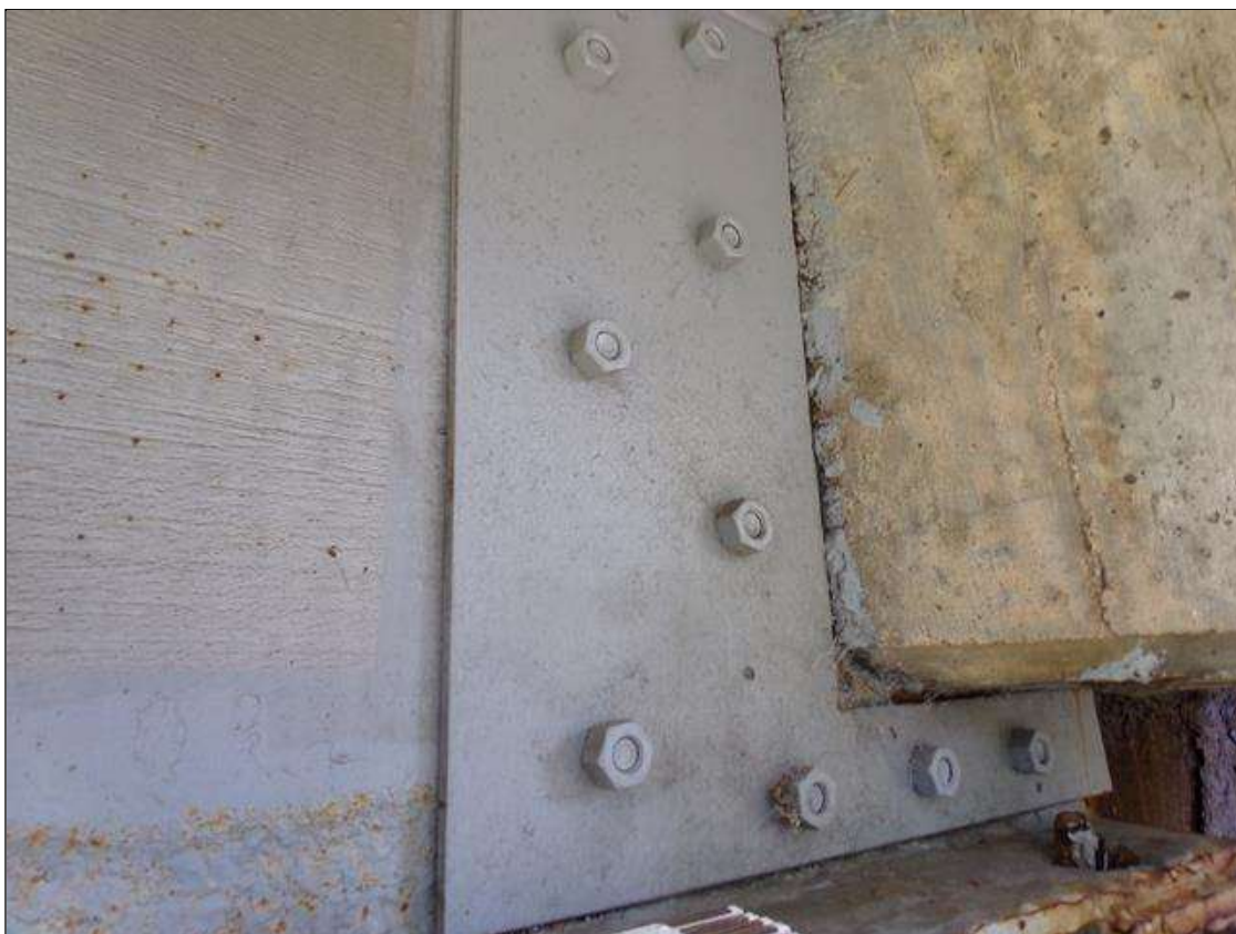
BOLTED PLATE REPAIR FULL HEIGHT X 1' LONG TO WEB AT BENT 3 BEAM 1 SPAN 4
