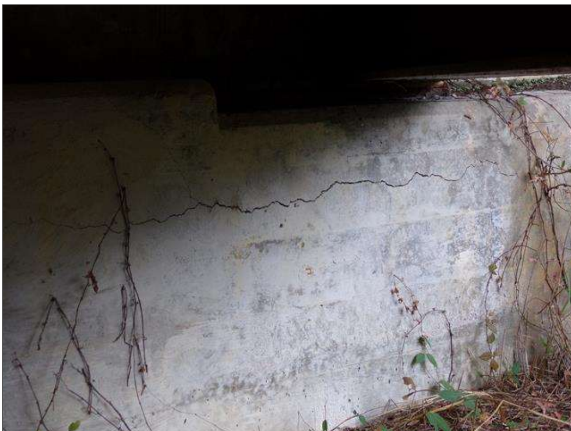
End Bent 2 Cap 1: HORIZONTAL CRACK 4 FT LONG UP TO 1/8" WIDE IN FACE OF CAP UNDER BEAM 5
