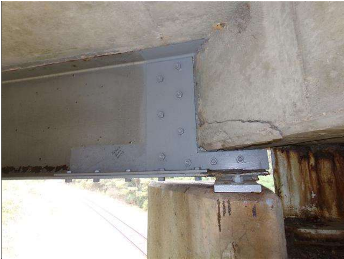
BOLTED PLATE REPAIR 24" X 24" TO WEB BOTH SIDES AND 24" BOTTOM FLANGE WEST SIDE BEAM 5 SPAN 4 AT BENT 3
