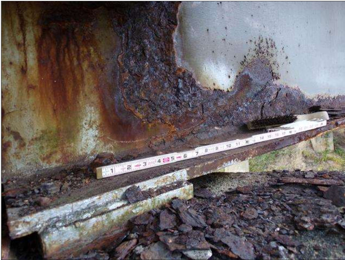
Span 3 Beam 5: 4 FT. OF ACTIVE CORROSION WITH 1/2" REMAINING SECTION IN WEB AROUND DIAPHRAM AND BOTTOM 6" OF WEB AND 3/4" THICKNESS REMAINING FULL WIDTH BOTTOM FLANGE AT BENT 2 BEAM ENDS HAVE BEEN PAINTED WITH ACTIVE SURFACE CORROSION
