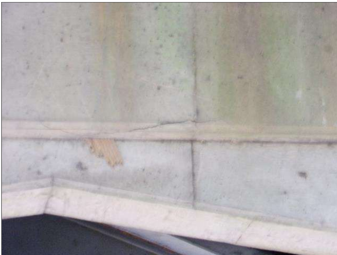
Bent 2 Cap 1: 3 FT X 1.5 FT HIGH DELAMINATION WITH CRACK UP TO 1/4" WIDE IN SOUTH FACE UNDER BEAM
