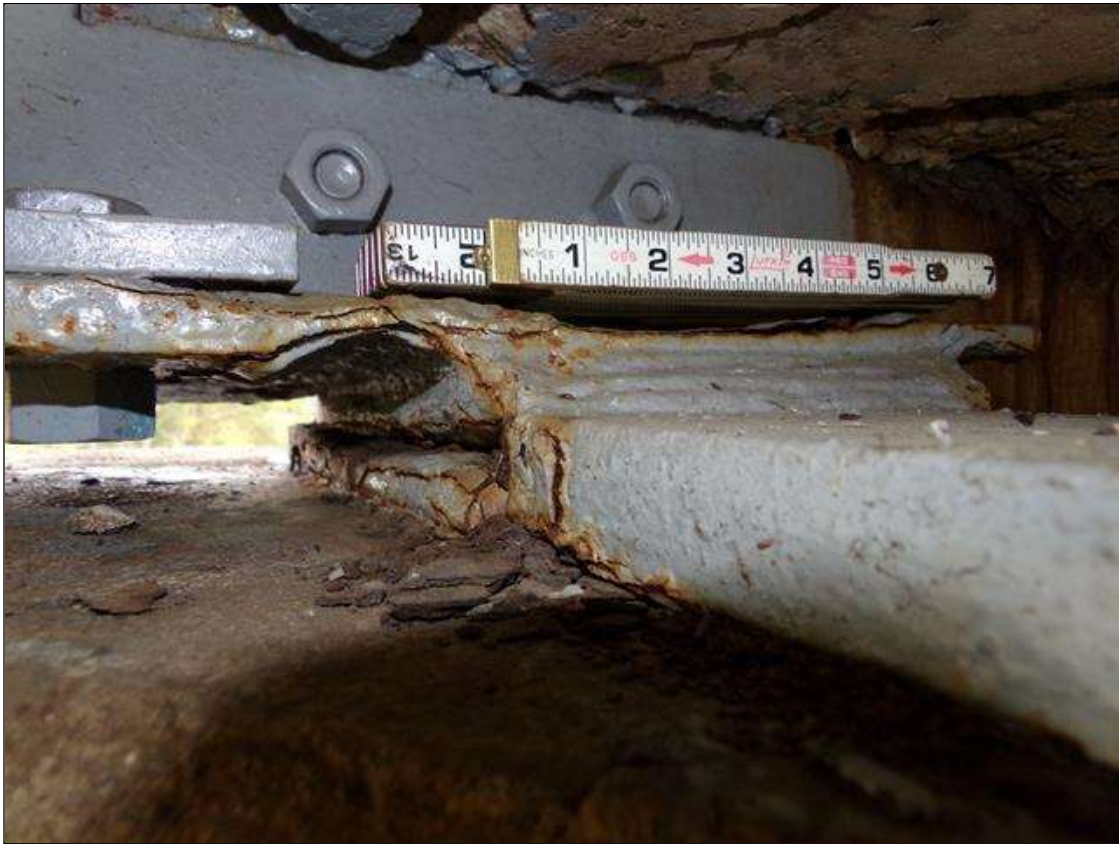
Span 4 Beam 5: PAR--SECTION LOSS UP TO 3/8" WITH 3/8" AVERAGE REMAINING FULL WIDTH OF BOTTOM FLANGE 1FT LONG ON BEAM END OVER PIER 3. BEAM END HAS BEEN CLEANED AND PAINTED WITH ACTIVE SURFACE CORROSION. PLATE REPAIR ADDED BUT DOES NOT EXTEND OUT TO DEFECT.
