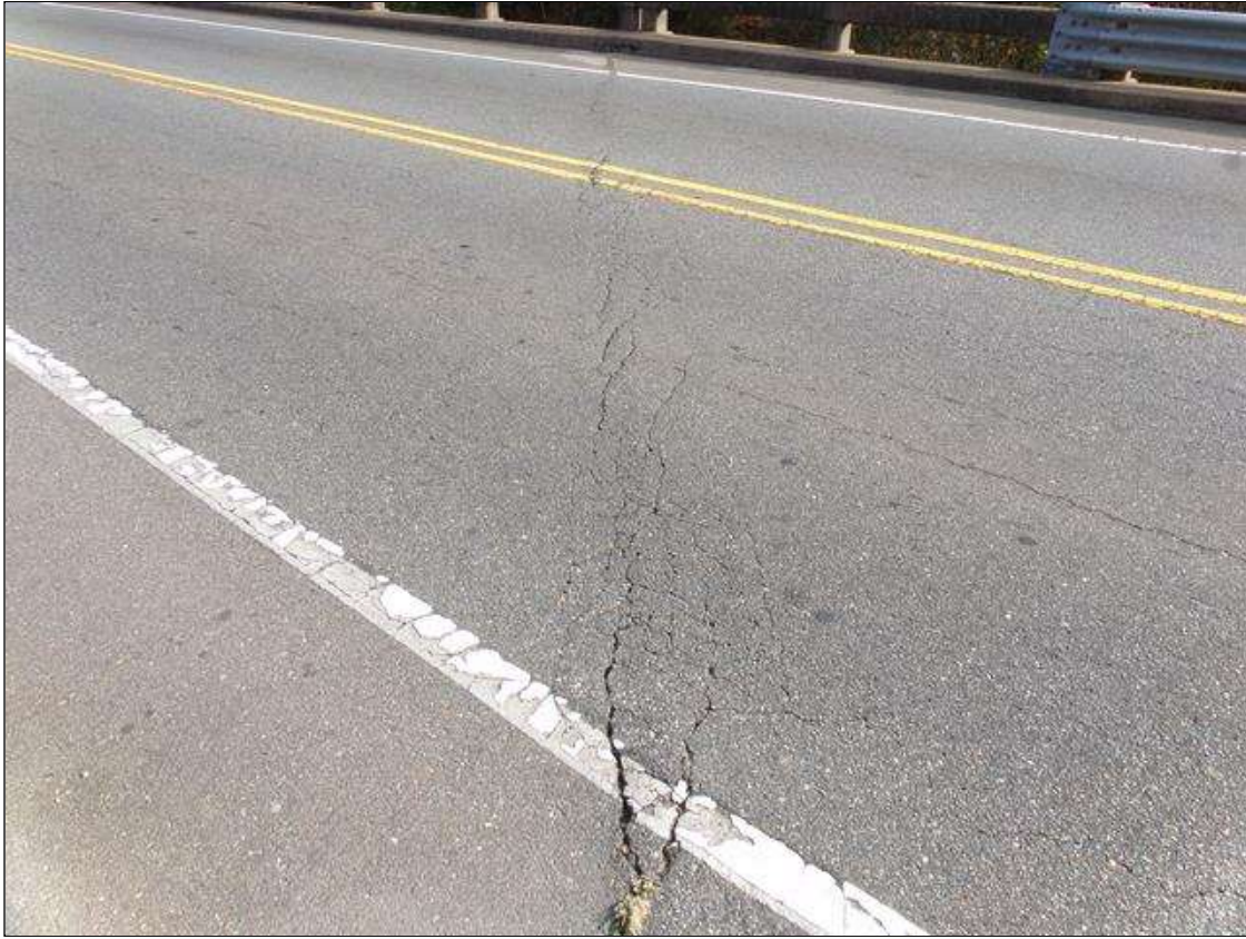
Span 1 Wearing Surface: FULL WIDTH TRANSVERSE/MAP CRACKING UP TO 1/2" WIDE OVER END BENT 1 AND BENT 1, BENT 1 SHOWN
