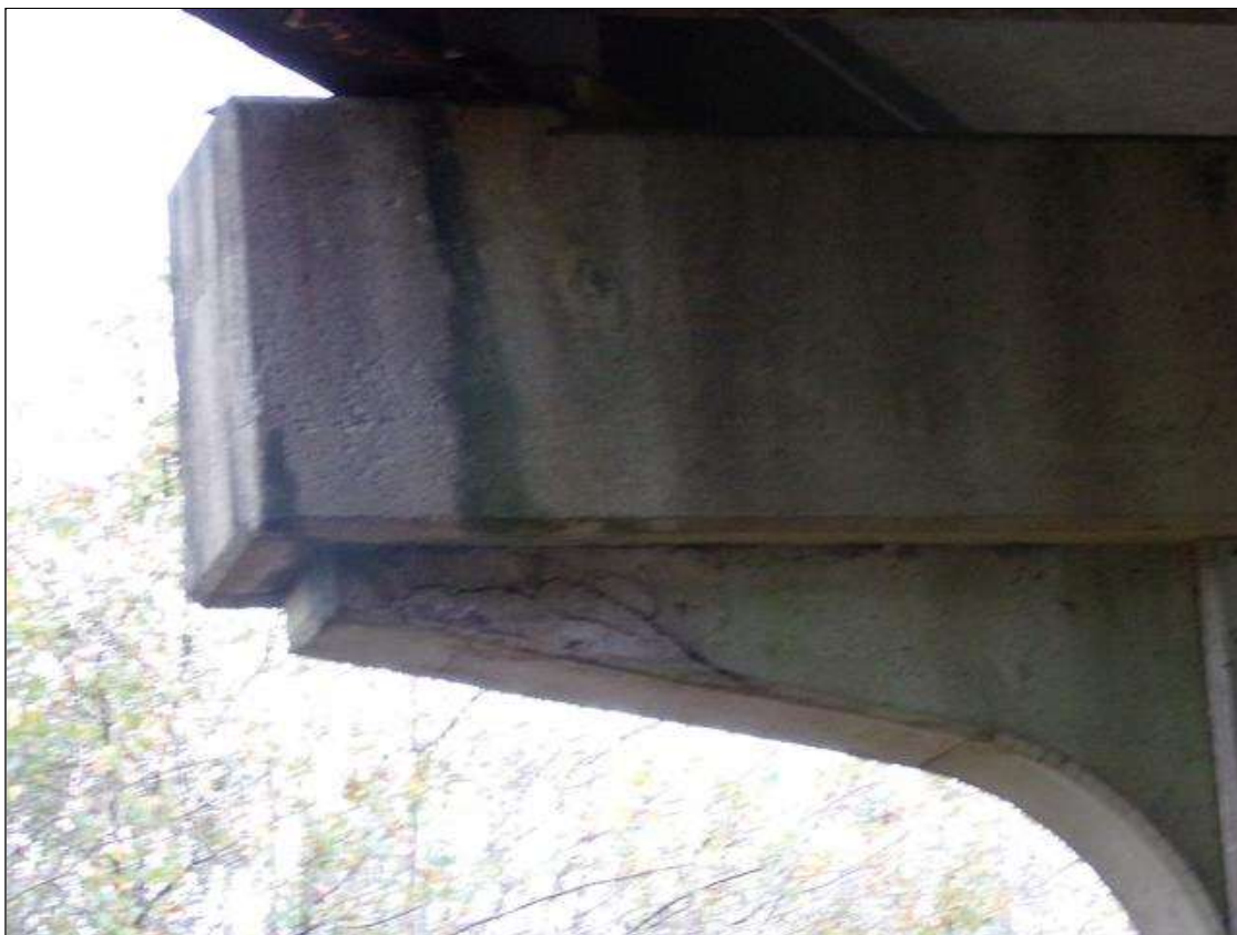
Bent 2 Cap 1: 3 FT X 1 FT X 6" DELAMINATION IN UNDERSIDE UNDER BEAM 5 IN FLUTED PORTION
