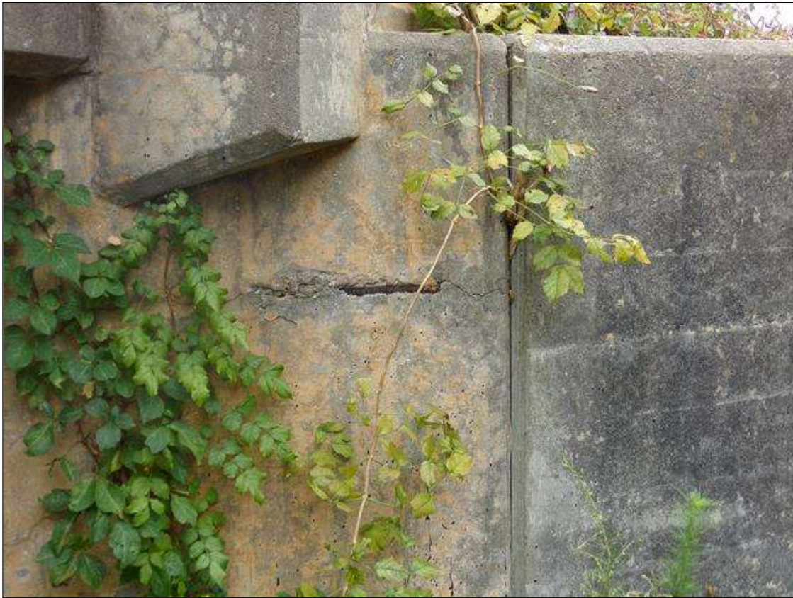
End Bent 1 Abutment/Backwall : SPALL WITH EXPOSED REBAR 12" X 2" X 1/2" DEEP WITH CRACK WITH EFFLORESCENCE 12" LONG X UP TO 1/32" WIDE IN CURTAIN WALL AT WEST END
