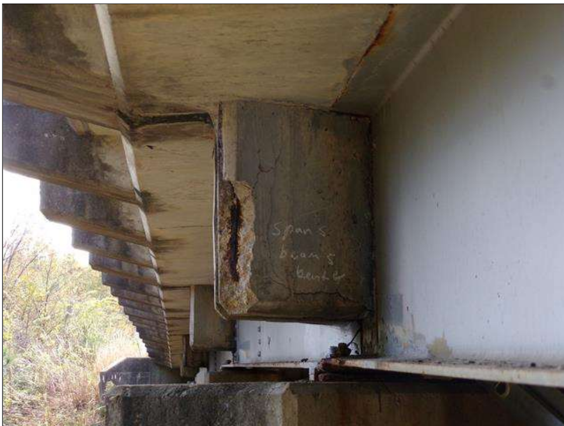
12" X 4" X 2" DEEP SPALL WITH EXPOSED REBAR IN BENT 4 END DIAPHRAGM AT EAST END
