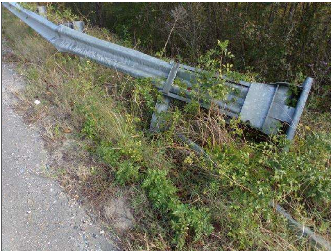
Guardrail impact damage to southeast terminal end
