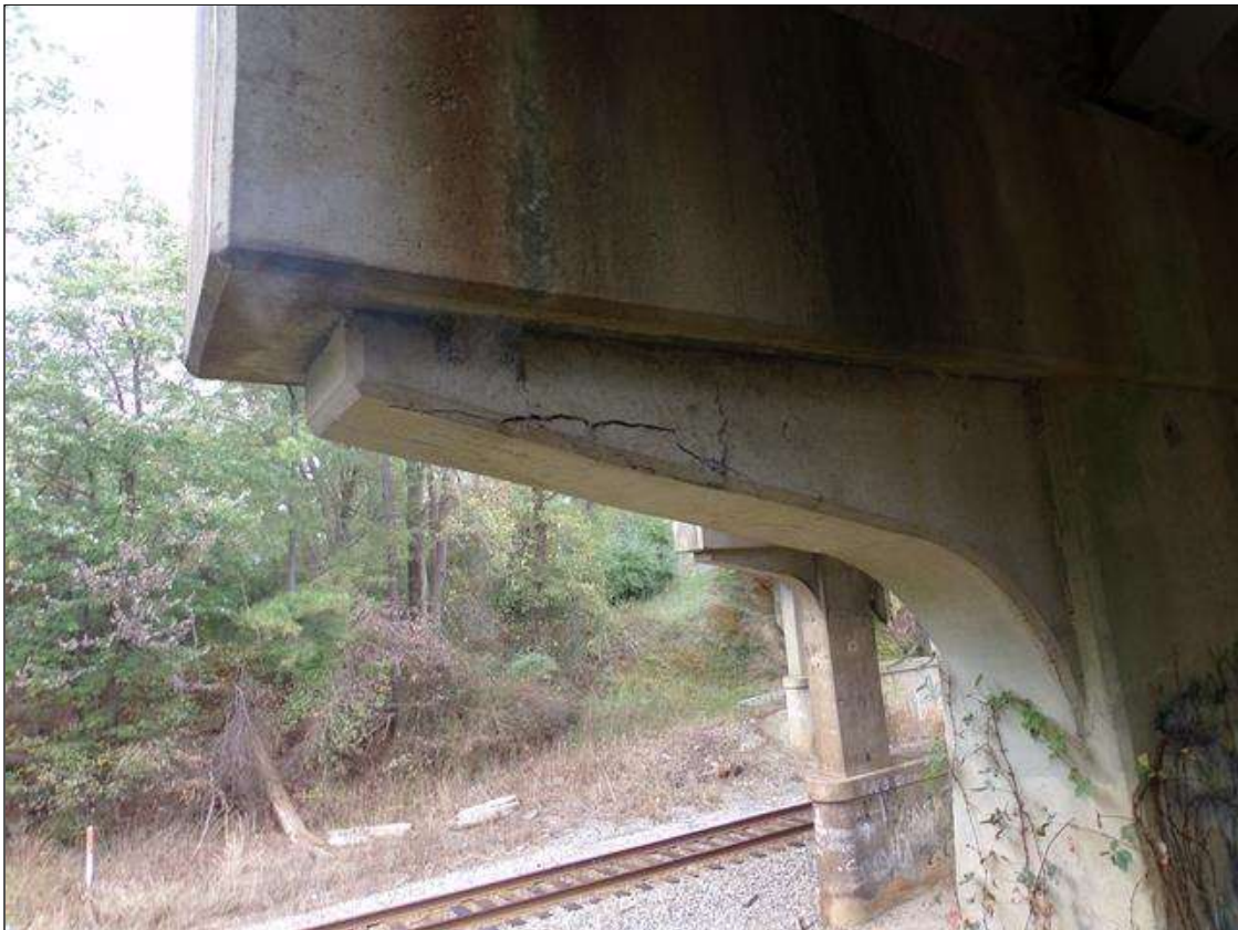
Bent 1 Cap 1: 24" X 8" DELAMINATION WITH CRACKS UP TO 1/4" WIDE IN SOUTH FACE UNDER WEST OVERHANG IN FLUTED PORTION
