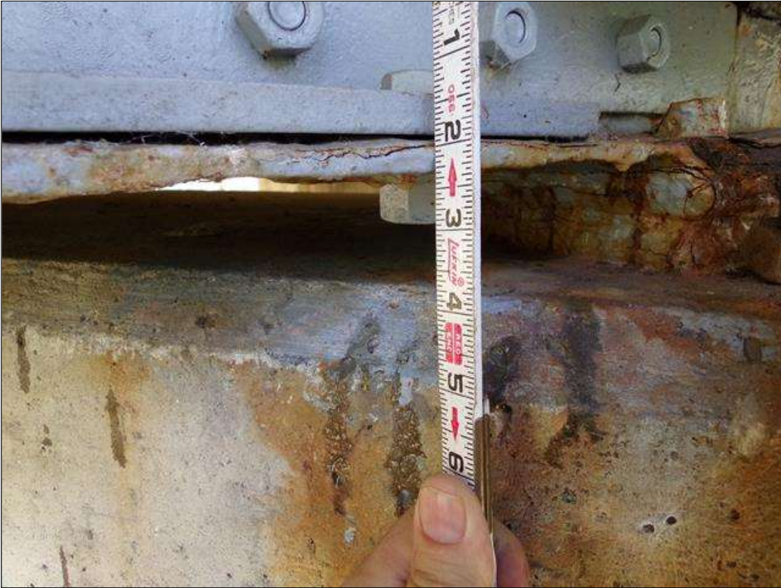
Span 5 Beam 1: 1/4" section loss with 3/8" average remaining full width of bottom flange. Beam end has been painted with active surface corrosion present. No PAR issued due to repair plate added at pier 4.
