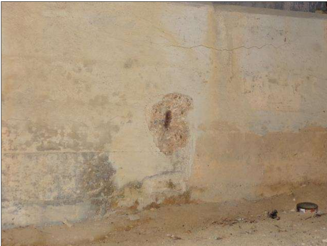
End Bent 1 Cap 1: 8" DIAMETER X 1" DEEP SPALL WITH EXPOSED REBAR UNDER BAY 4
