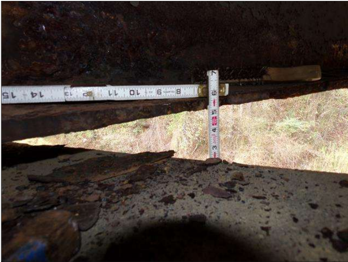
Span 3 Beam 1: PAR--SECTION LOSS WITH 7/16" REMAINING SECTION IN WEB AROUND END DIAPHRAGM 1 FT LONG AND 1/2" REMAINING IN BOTTOM 6" OF WEB WITH 5/8" X FULL WIDTH REMAINING 3 FT LONG ON BOTTOM FLANGE AT BENT 2
