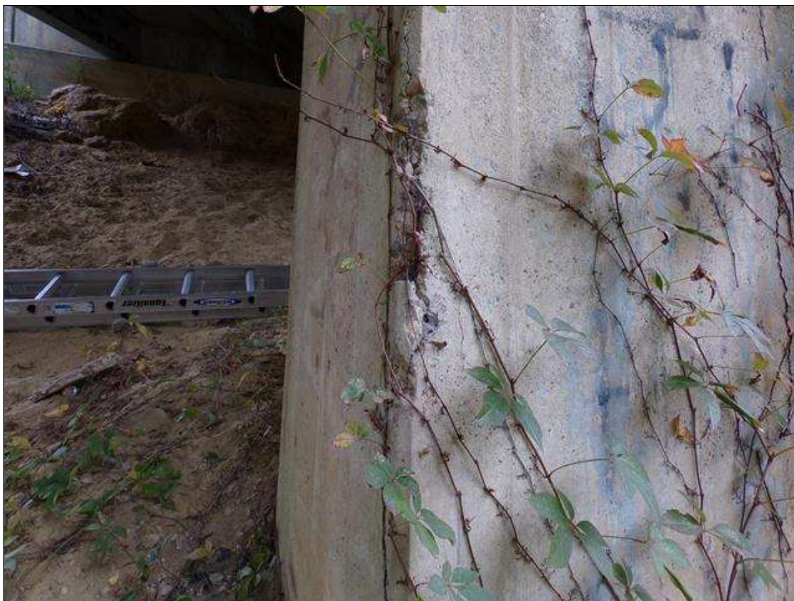
Bent 1 Pile 1: 3 FT X 9" X 1" DEEP SPALL AND DELAMINATION AT NORTHEAST CORNER
