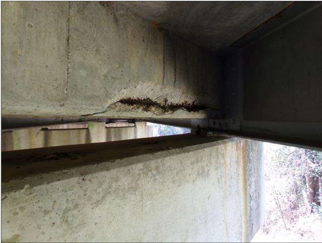
36" X 8" X 3" DEEP SPALL WITH EXPOSED REBAR IN BENT 4 END DIAPHRAGM IN BAY 1 SPAN 5 AND A 9" WIDE X 1' HIGH X 2" DEEP SPALL AT BEAM 2 IN BAY 1 SPAN 5
