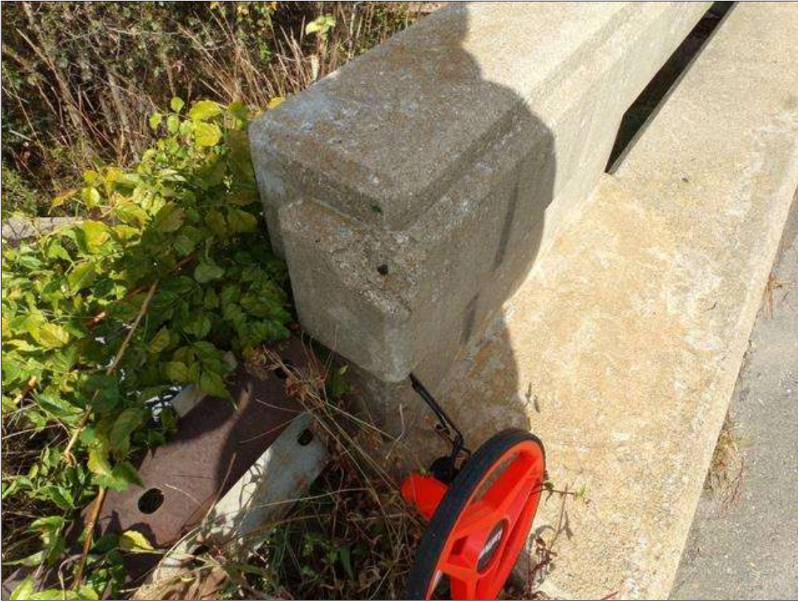
Span 1 Left Bridge Rail: 4" DIAMETER X 1" DEEP SPALL WITH EXPOSED REBAR AT END POST AT SOUTHWEST CORNER
