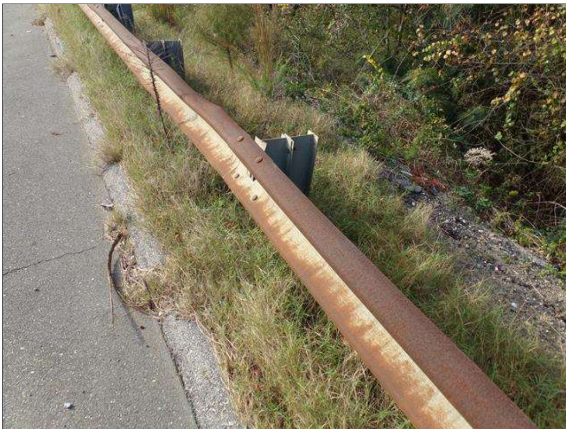
Guardrail impact damage to southwest rail 40' from bridge 10' long
