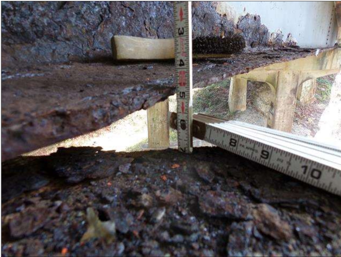
Span 3 Beam 1: PAR--CORROSION 5FT LONG WITH UP TO 5/8" LOSS AT OUTER EDGES OF BOTTOM FLANGE WITH 1/2" AVERAGE REMAINING FULL WIDTH AND 1/2" THICKNESS REMAINING IN WEB 5FT LONG AT BENT 3
