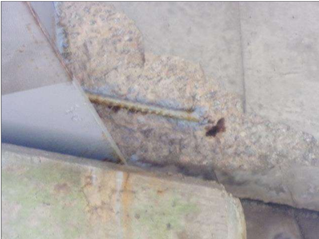
18" X 12" X 3" DEEP SPALL WITH EXPOSED REBAR AND A 1' LONG X 9" WIDE X 2" DEEP SPALL NO EXPOSED REBAR AT BEAM 2 IN BENT 3 DIAPHRAGM OVER PIER 3 IN BAY 1, BAY 2 SIMILAR
