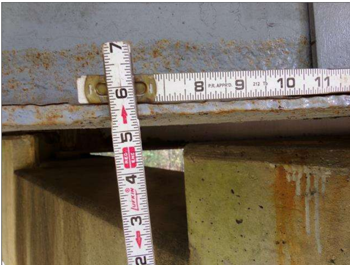
Span 4 Beam 1: PAR--1/4" section loss with 3/8" average remaining full width of bottom flange 3' long. Beam end has been painted with rust staining present at pier 3.
