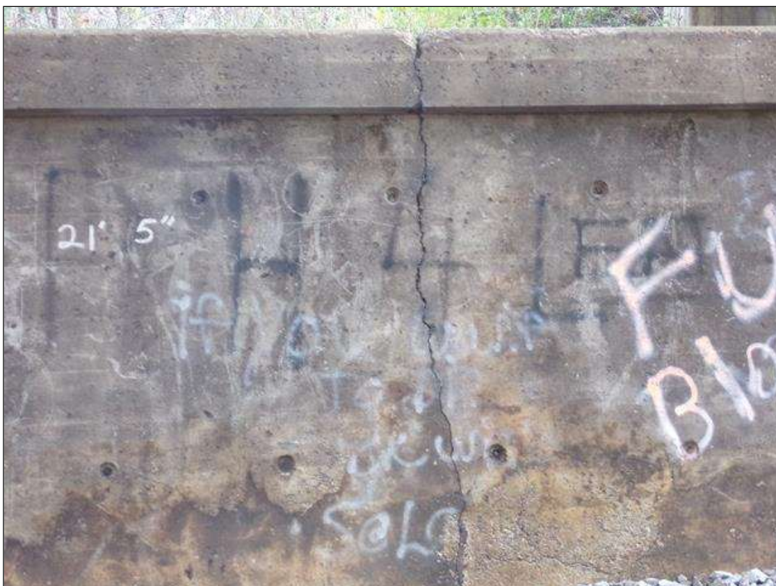
Bent 2 Pile 1: VERTICAL THRU CRACK 7 FT LONG UP TO 1/2" WIDE IN MIDDLE OF CRASH WALL BOTH FACES
