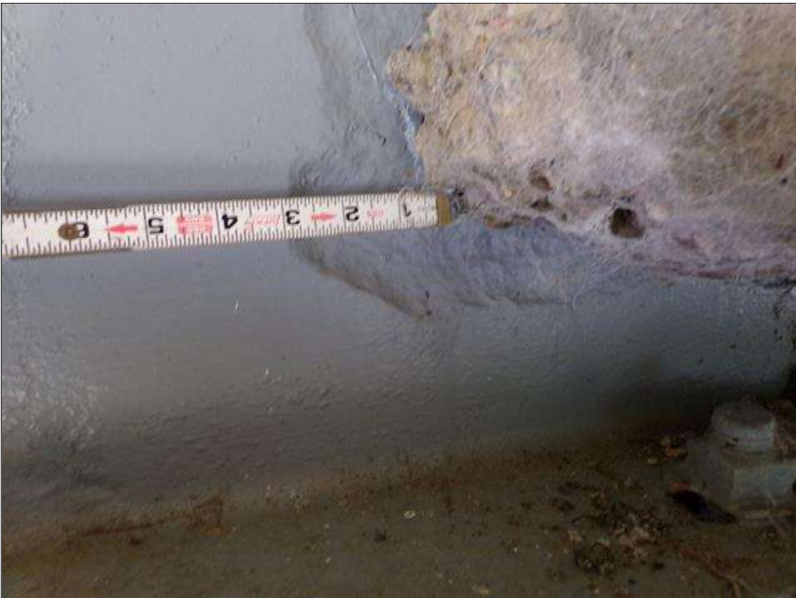
Span 5 Beam 2: PAR--1 FT LONG X 2" WIDE AREA OF PREVIOUS CORROSION WITH 1/4" REMAINING SECTION IN WEB AROUND END DIAPHRAGM AT BENT 4 AREA HAS BEEN PAINTED OVER AND ARRESTED.
