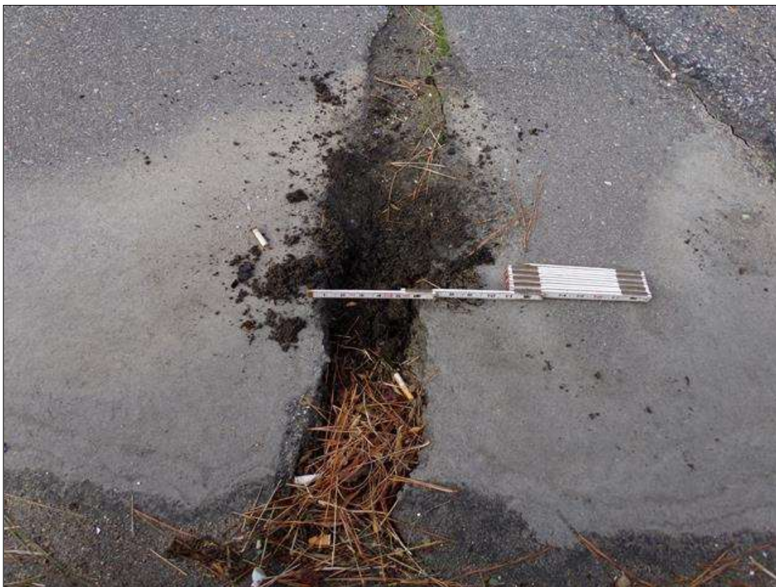
Span 3 Wearing Surface: 3' Long x 6" wide x 2 1/2" deep pothole at right shoulder at pier 3
