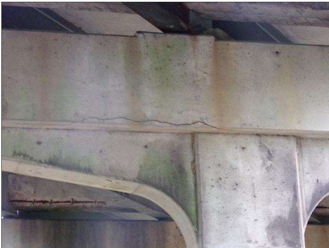
Bent 2 Cap 1: 6FT LONG HORIZONTAL CRACK UP TO 1/4" WIDE UNDER BAYS 1 AND 2 NORTH FACE
