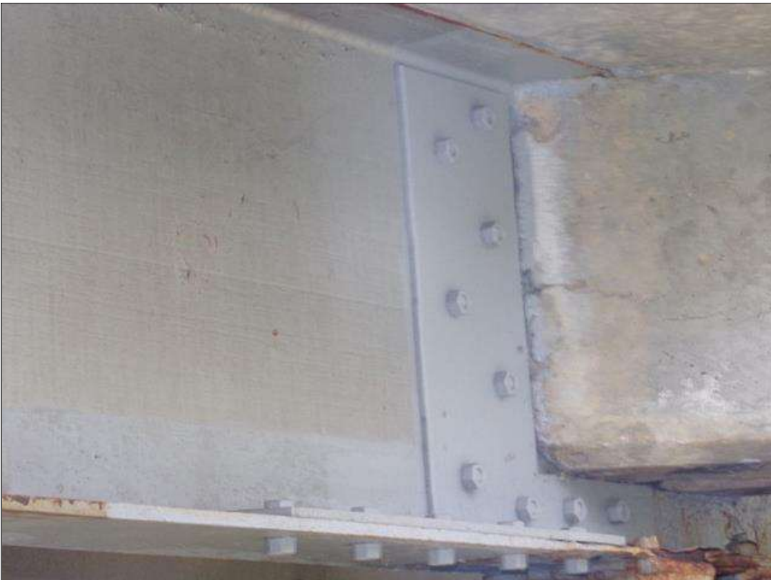
BEAM 1 BOLTED PLATE REPAIR TO BOTTOM FLANGE WEST SIDE AND BOTH FACES OF WEB AT BENT 4 SPAN
