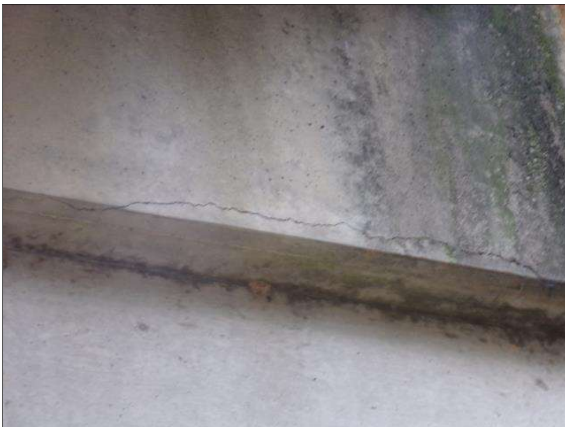
Bent 1 Cap 1: 6' LONG X 1/8" WIDE HORIZONTAL CRACK NORTH FACE UNDER BAY 1
