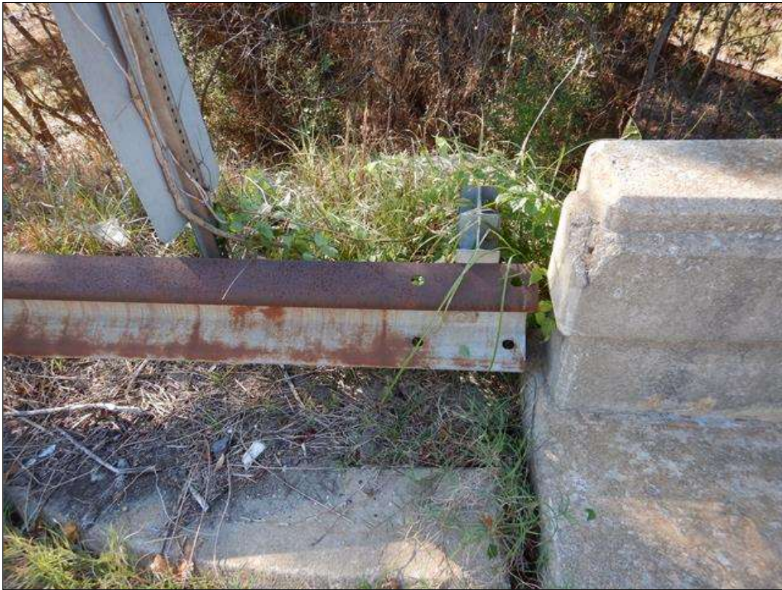
SOUTHWEST CORNER, GUARDRAIL NOT CONNECTED
