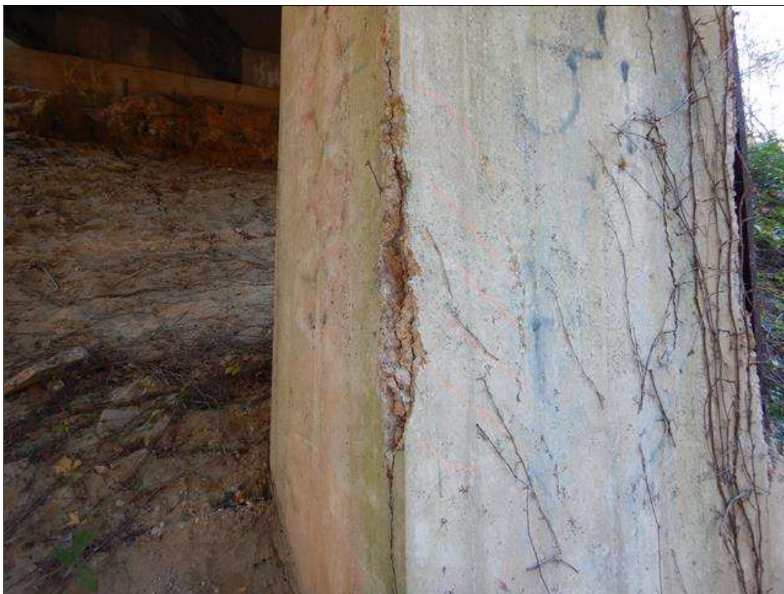
Bent 1 Pile 1: 3 FOOT X 9" X 1" DEEP SPALL AND DELAMINATION AT NORTHEAST CORNER
