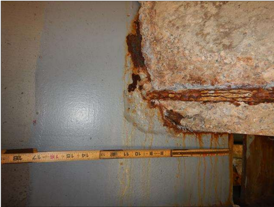
Span 2 Beam 2: [PROMPT ACTION REQUEST] BEAM END AT BENT 1 AT THE INTERFACE WITH THE REINFORCED CONCRETE DIAPHRAGM, THERE IS A BAND OF CORROSION UP TO 3" WIDE WITH SECTION LOSS [AVERAGE 3/8" REMAINS] FOR APPROXIMATELY 1' LONG X UP TO THE FULL HEIGHT OF THE DIAPHRAGM.
