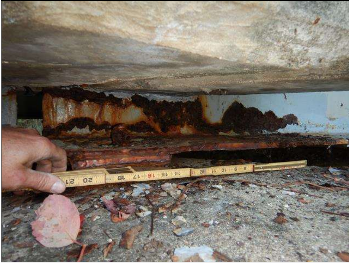
Span 5 Beam 5: [PROMPT ACTION REQUEST] BEAM END AT BENT 4 IN THE LOWER FLANGE, CORROSION WITH SECTION LOSS [AVERAGE 1/4" REMAINS] FOR APPROXIMATELY 4' LONG. AT THE SAME END IN THE LOWER 4" OF THE WEB, CORROSION WITH SECTION LOSS [AVERAGE 5/16" REMAINS] FOR APPROXIMATELY 4' LONG.
