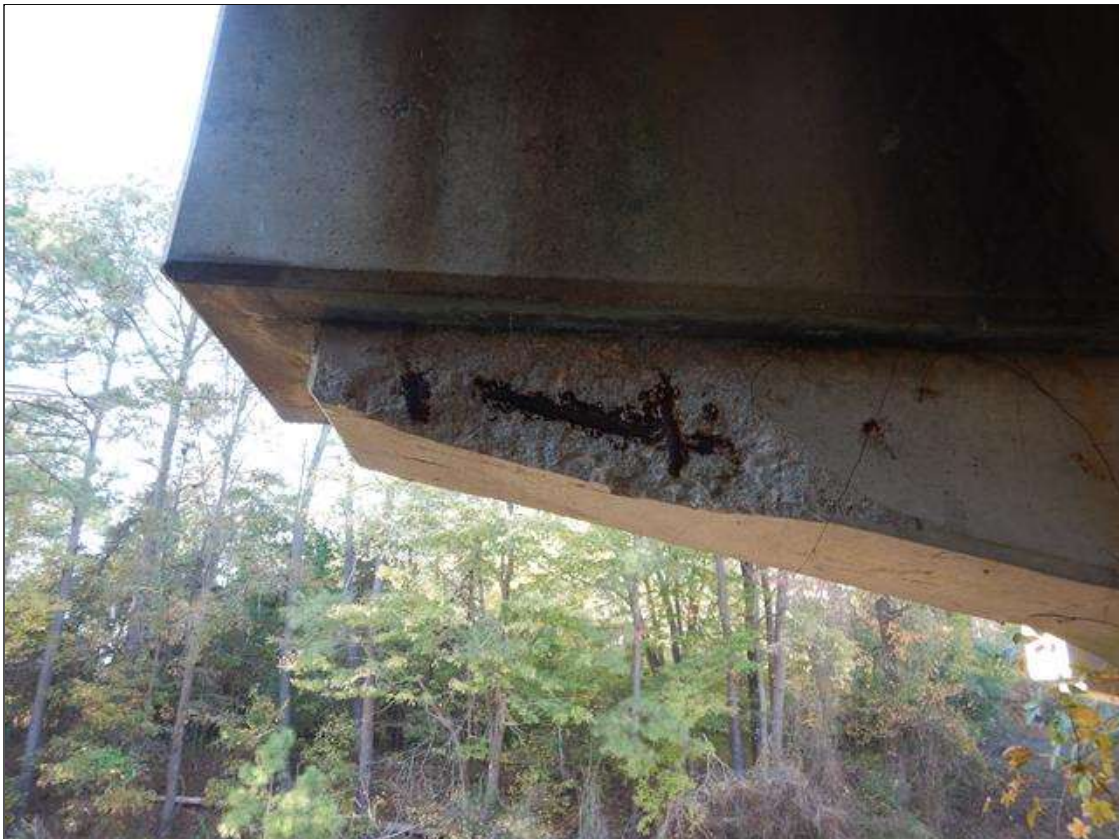
Bent 1 Cap 1: [PROMPT ACTION REQUEST] SOUTH FACE AT THE LEFT END, LOWER 10", SPALLING WITH EXPOSED REBAR [APPROXIMATELY 40" LONG X UP TO 2.5" DEEP]
