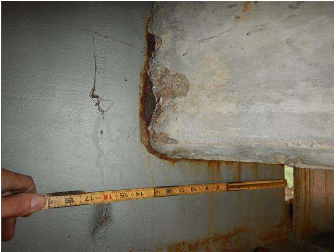
Span 1 Beam 2: [PROMPT ACTION REQUEST] BEAM END AT BENT 1 AT THE INTERFACE WITH THE REINFORCED CONCRETE DIAPHRAGM, THERE IS A BAND OF CORROSION UP TO 1" WIDE WITH SECTION LOSS [AVERAGE 3/8" REMAINS] FOR APPROXIMATELY 1' LONG X UP TO THE FULL HEIGHT OF THE DIAPHRAGM.
