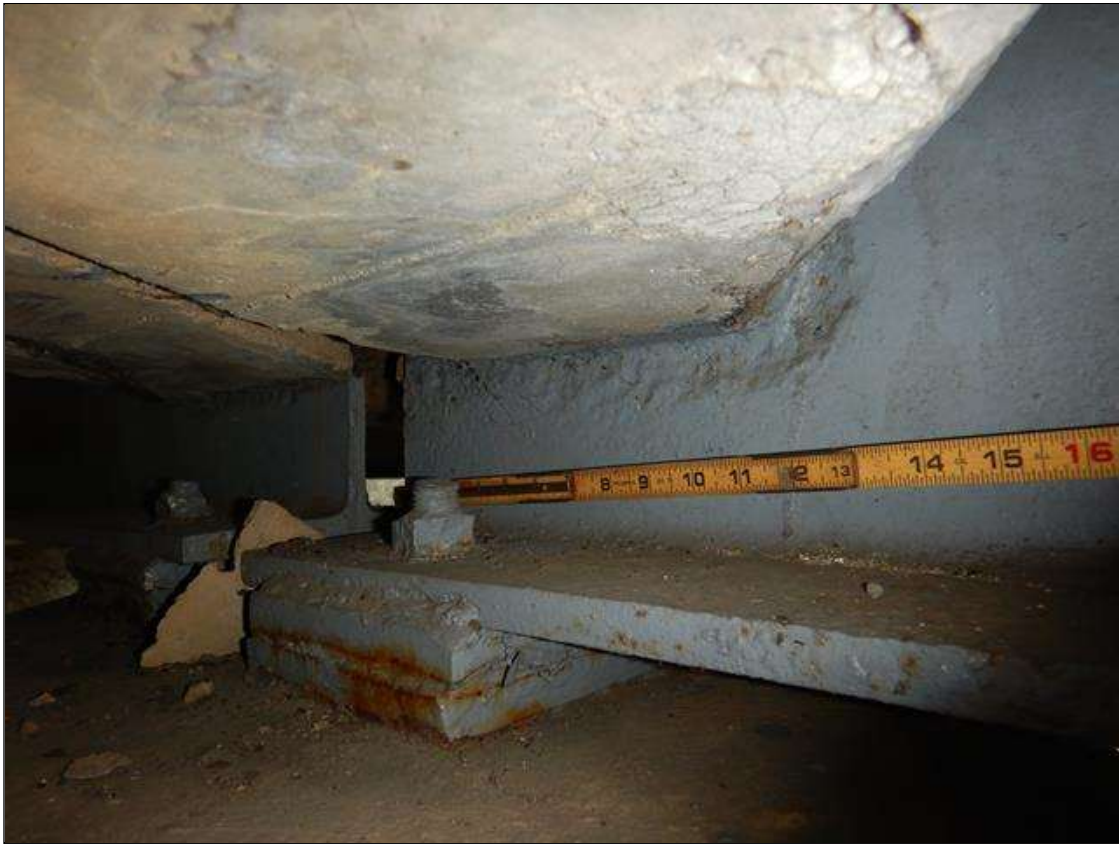
Span 4 Beam 3: [PROMPT ACTION REQUEST] BEAM END AT BENT 4 AT THE INTERFACE WITH THE REINFORCED CONCRETE DIAPHRAGM, THERE IS A BAND OF CORROSION UP TO 1" WIDE WITH SECTION LOSS [AVERAGE 5/16" REMAINS] FOR APPROXIMATELY 1' LONG X UP TO THE FULL HEIGHT OF THE DIAPHRAGM.
