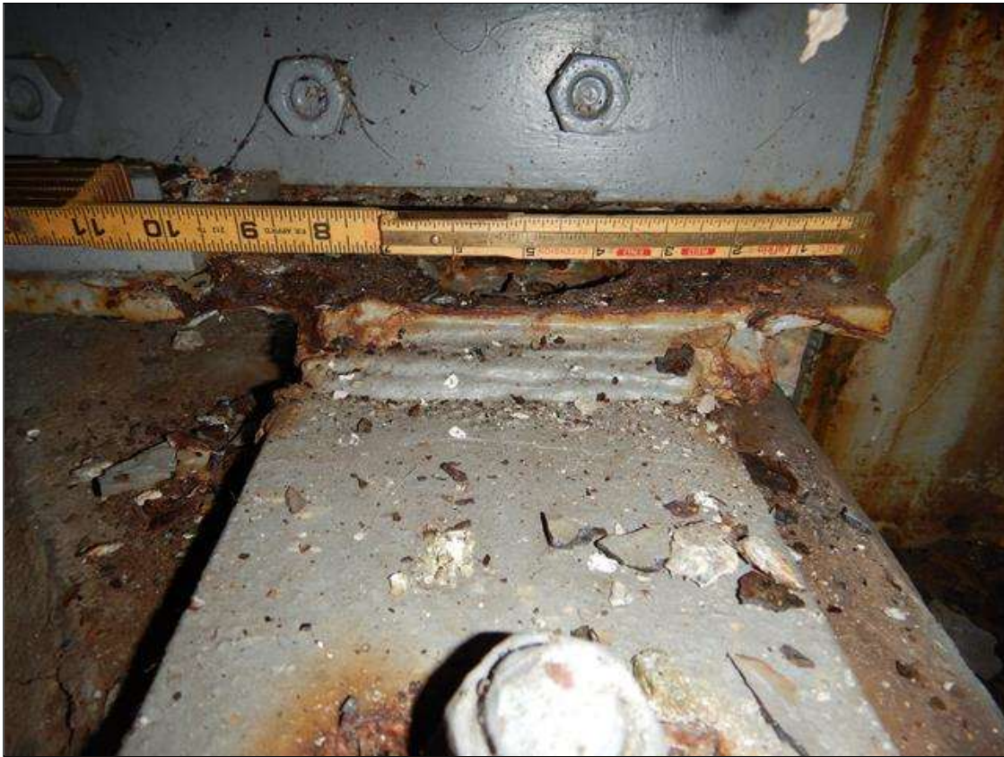
Span 4 Beam 5: PAR--SECTION LOSS UP TO 3/8" WITH 3/8" AVERAGE REMAINING FULL WIDTH OF BOTTOM FLANGE 1FT LONG ON BEAM END OVER PIER 3. BEAM END HAS BEEN CLEANED AND PAINTED WITH ACTIVE SURFACE CORROSION. PLATE REPAIR ADDED BUT DOES NOT EXTEND OUT TO DEFECT.
