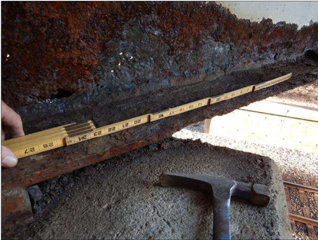
Span 3 Beam 1: [PROMPT ACTION REQUEST] BEAM END AT BENT 3 IN THE LEFT LOWER FLANGE, CORROSION WITH SECTION LOSS [AVERAGE 1/16" REMAINS] FOR APPROXIMATELY 4' LONG WITH EDGE HOLES UP TO 3/4" DIAMETER. AT THE SAME END IN THE LOWER 6" OF THE WEB, CORROSION WITH SECTION LOSS [AVERAGE 1/16" REMAINS] FOR APPROXIMATELY 4' LONG WITH PERFORATIONS THROUGHOUT.
