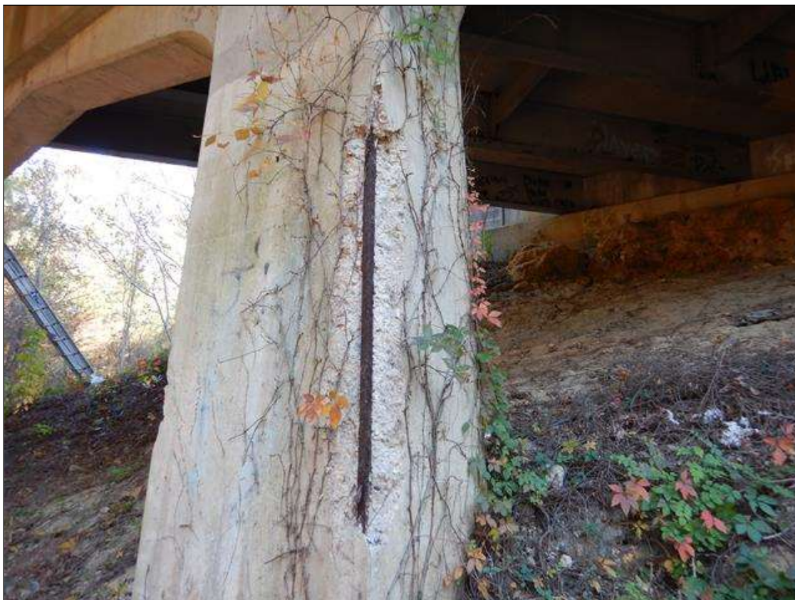
Bent 1 Pile 1: [PROMPT ACTION REQUEST] 6 FOOT X 9" X 2" DEEP SPALL WITH EXPOSED RUSTED REBAR NO SECTION LOSS AT NORTHWEST CORNER
