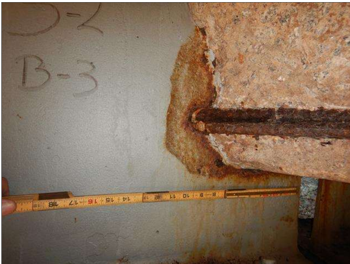
Span 2 Beam 3: [PROMPT ACTION REQUEST] BEAM END AT BENT 1 AT THE INTERFACE WITH THE REINFORCED CONCRETE DIAPHRAGM, THERE IS A BAND OF CORROSION UP TO 3" WIDE WITH SECTION LOSS [AVERAGE 3/8" REMAINS] FOR APPROXIMATELY 1' LONG X UP TO THE FULL HEIGHT OF THE DIAPHRAGM.
