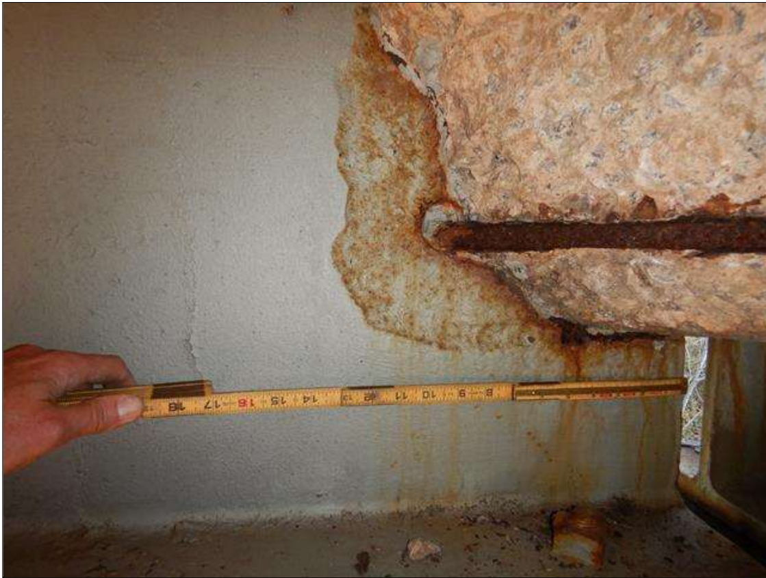
Span 2 Beam 5: [PROMPT ACTION REQUEST] BEAM END AT BENT 1 AT THE INTERFACE WITH THE REINFORCED CONCRETE DIAPHRAGM, THERE IS A BAND OF CORROSION UP TO 3" WIDE WITH SECTION LOSS [AVERAGE 3/8" REMAINS] FOR APPROXIMATELY 1' LONG X UP TO THE FULL HEIGHT OF THE DIAPHRAGM.
