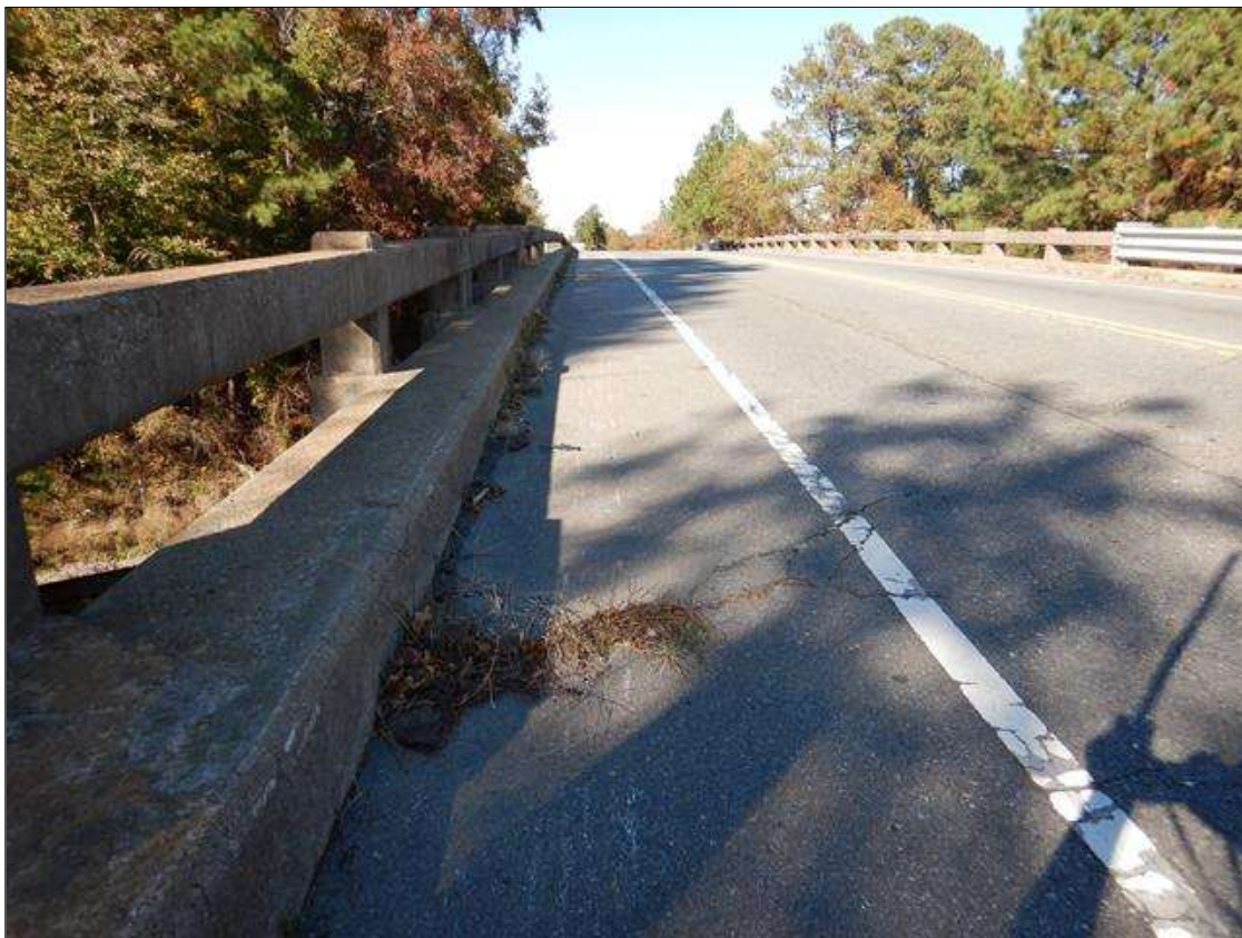
RIGHT AND LEFT GUTTERLINES, DEBRIS ACCUMULATION ALONG THE LENGTHS
