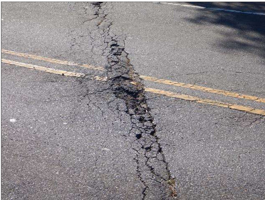
Span 3 Wearing Surface: FULL WIDTH TRANSVERSE/MAP CRACK UP TO 2" WIDE WITH ASPHALT DETERIORATION WITH UP TO 3/4" DEEP POT HOLES UP TO 1' LONG X 2" WIDE OVER BENT 3
