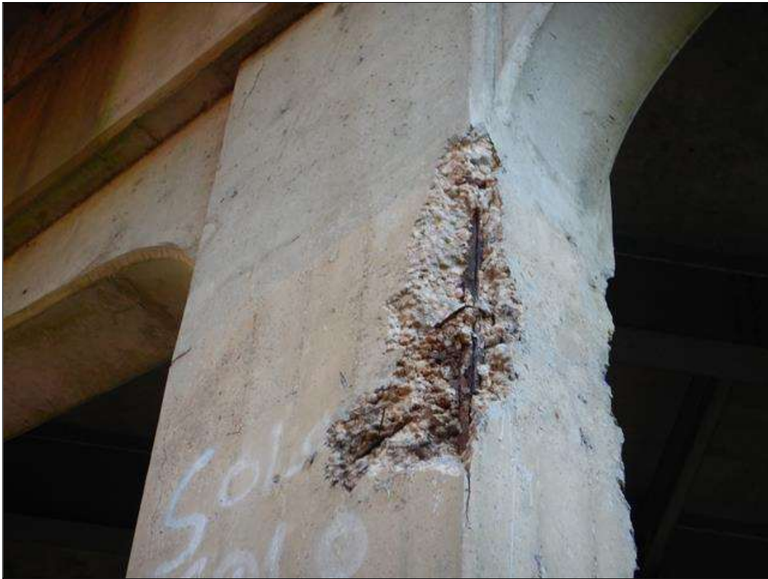
Bent 3 Pile 2: [PROMPT ACTION REQUEST] NORTHEAST CORNER, SPALLING WITH EXPOSED REBAR [APPROXIMATELY 4' HIGH X UP TO 1.25' WIDE X UP TO 3" DEEP]
