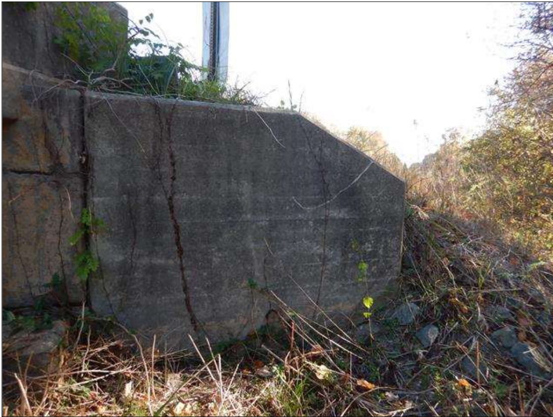
SOUTHWEST CORNER, REINFORCED CONCRETE WING [SIMILAR AT THE NORTHWEST CORNER, NORTHEAST CORNER, & SOUTHEAST CORNER]
