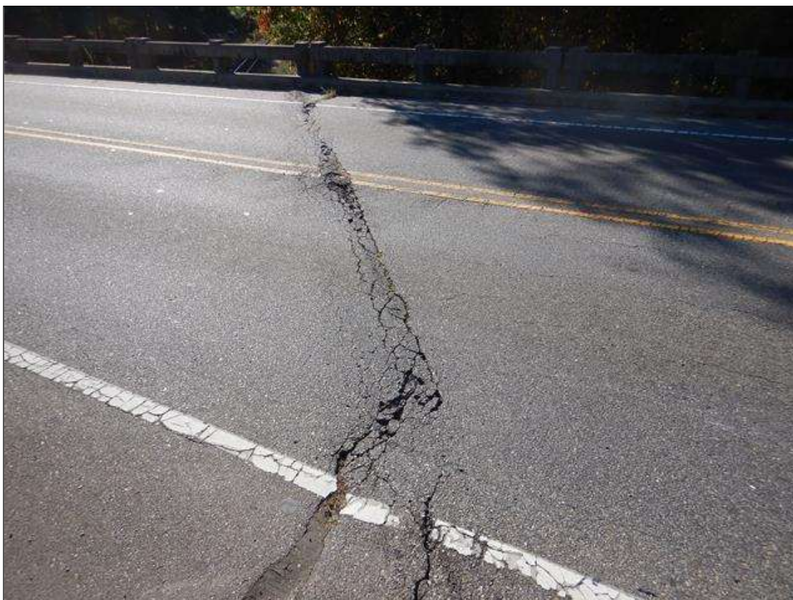
Span 3 Wearing Surface: FULL WIDTH TRANSVERSE/MAP CRACK UP TO 2" WIDE WITH ASPHALT DETERIORATION WITH UP TO 3/4" DEEP POT HOLES UP TO 1' LONG X 2" WIDE OVER BENT 3
