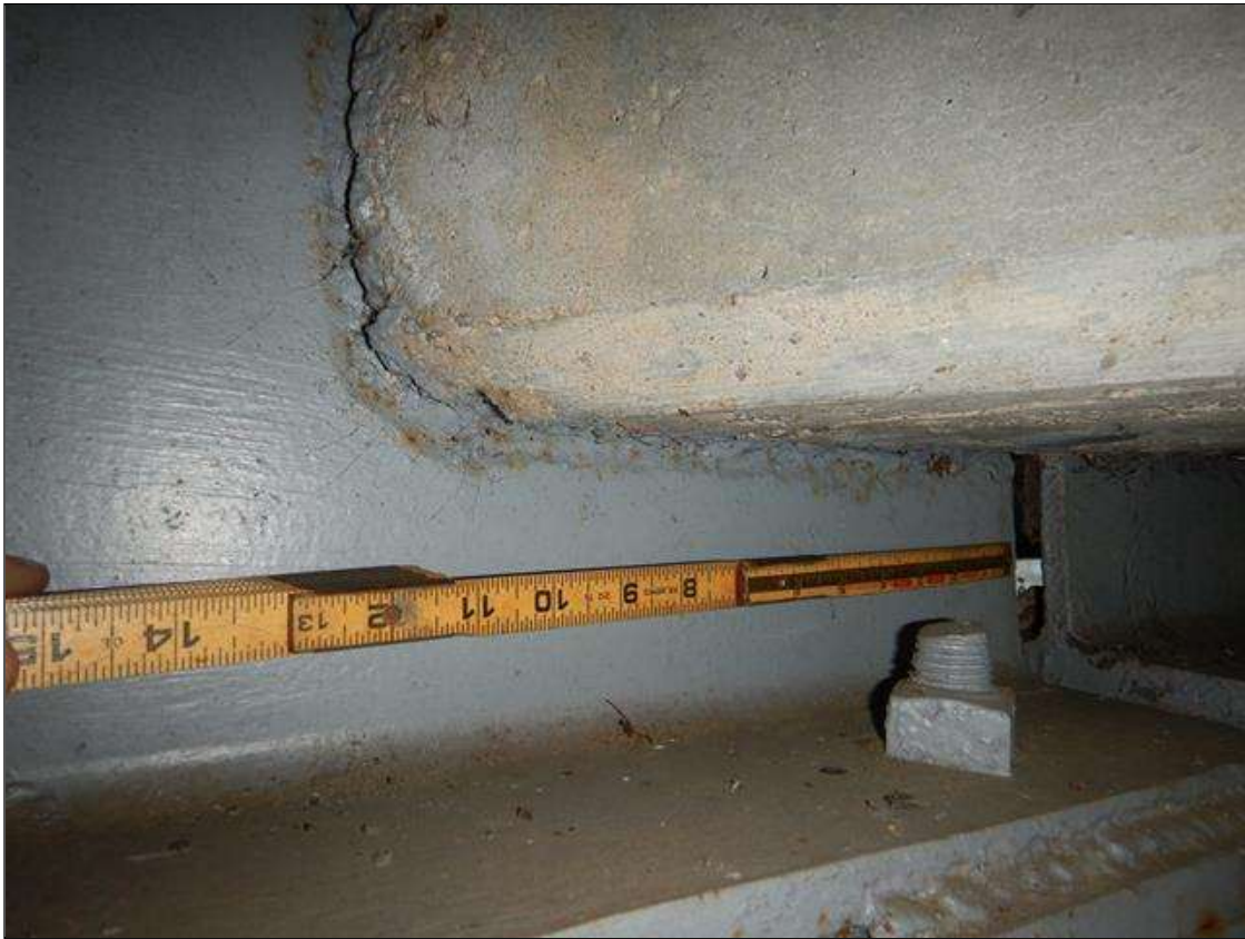
Span 4 Beam 2: [PROMPT ACTION REQUEST] BEAM END AT BENT 4 AT THE INTERFACE WITH THE REINFORCED CONCRETE DIAPHRAGM, THERE IS A BAND OF CORROSION UP TO 1" WIDE WITH SECTION LOSS [AVERAGE 3/8" REMAINS] FOR APPROXIMATELY 1' LONG X UP TO THE FULL HEIGHT OF THE DIAPHRAGM.
