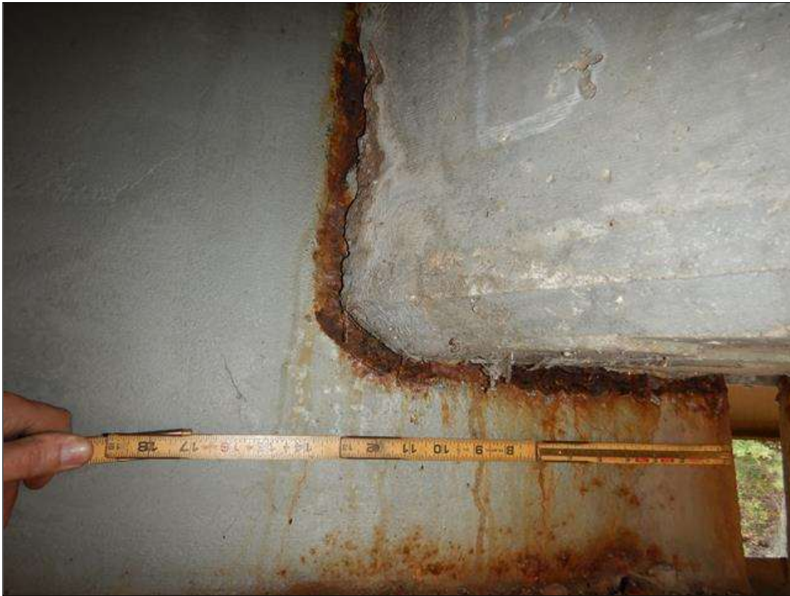
Span 1 Beam 3: [PROMPT ACTION REQUEST] BEAM END AT BENT 1 AT THE INTERFACE WITH THE REINFORCED CONCRETE DIAPHRAGM, THERE IS A BAND OF CORROSION UP TO 1" WIDE WITH SECTION LOSS [AVERAGE 3/8" REMAINS] FOR APPROXIMATELY 1' LONG X UP TO THE FULL HEIGHT OF THE DIAPHRAGM.
