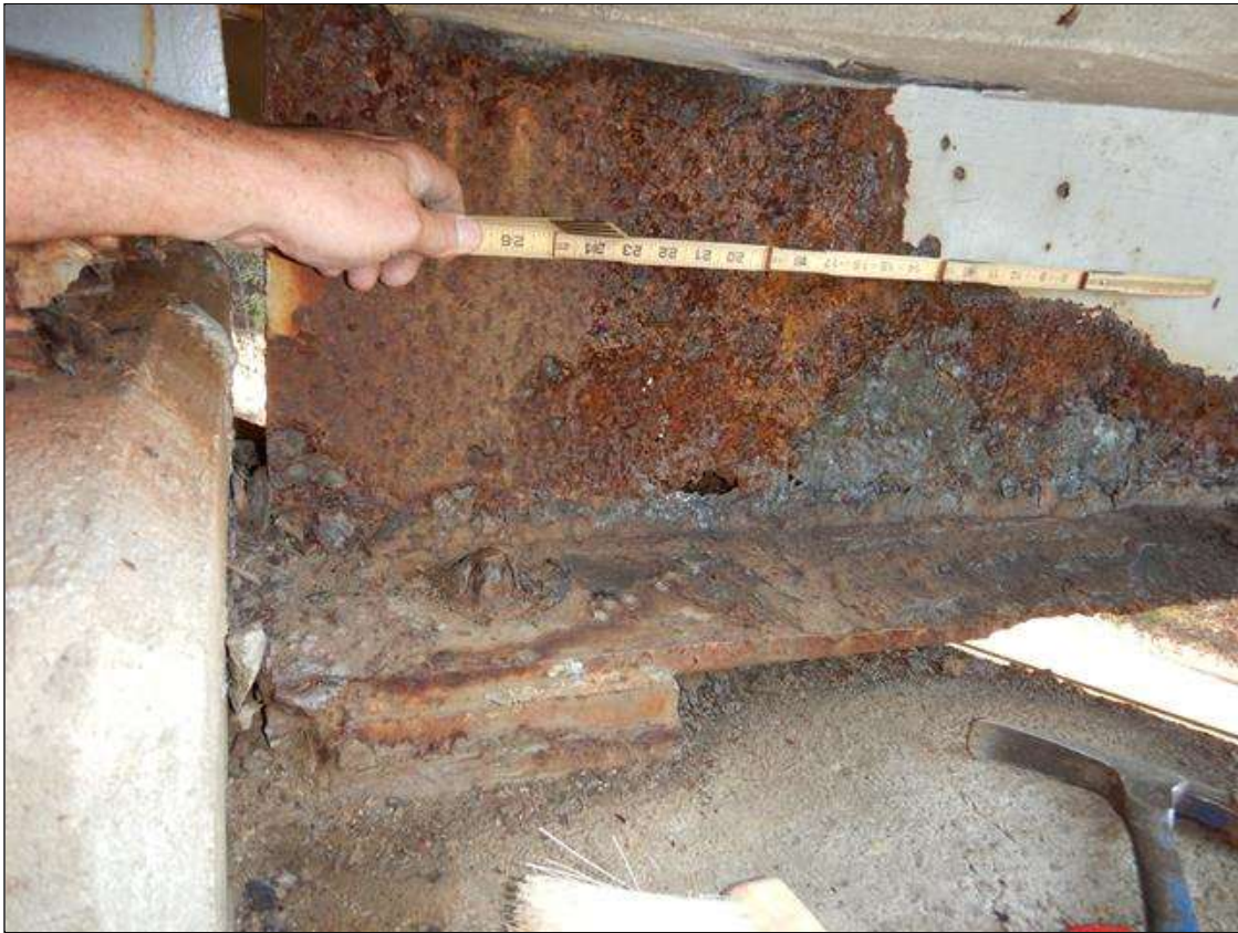
Span 3 Beam 1: [PROMPT ACTION REQUEST] BEAM END AT BENT 3 IN THE LEFT LOWER FLANGE, CORROSION WITH SECTION LOSS [AVERAGE 1/16" REMAINS] FOR APPROXIMATELY 4' LONG WITH EDGE HOLES UP TO 3/4" DIAMETER. AT THE SAME END IN THE LOWER 6" OF THE WEB, CORROSION WITH SECTION LOSS [AVERAGE 1/16" REMAINS] FOR APPROXIMATELY 4' LONG WITH PERFORATIONS THROUGHOUT.
