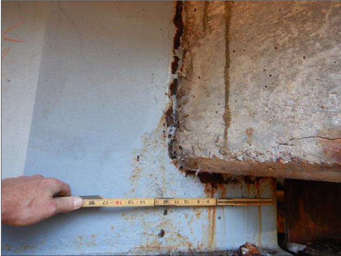
Span 2 Beam 1: [PROMPT ACTION REQUEST] BEAM END AT BENT 1 AT THE INTERFACE WITH THE REINFORCED CONCRETE DIAPHRAGM, THERE IS A BAND OF CORROSION UP TO 2" WIDE WITH SECTION LOSS [AVERAGE 3/8" REMAINS] FOR APPROXIMATELY 1' LONG X UP TO THE FULL HEIGHT OF THE DIAPHRAGM.
