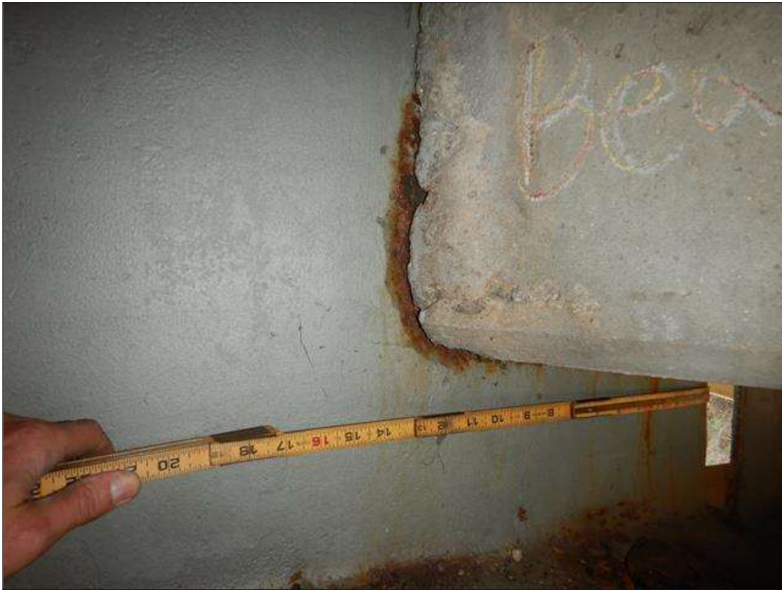
Span 1 Beam 4: [PROMPT ACTION REQUEST] BEAM END AT BENT 1 AT THE INTERFACE WITH THE REINFORCED CONCRETE DIAPHRAGM, THERE IS A BAND OF CORROSION UP TO 1" WIDE WITH SECTION LOSS [AVERAGE 3/8" REMAINS] FOR APPROXIMATELY 1' LONG X UP TO THE FULL HEIGHT OF THE DIAPHRAGM.
