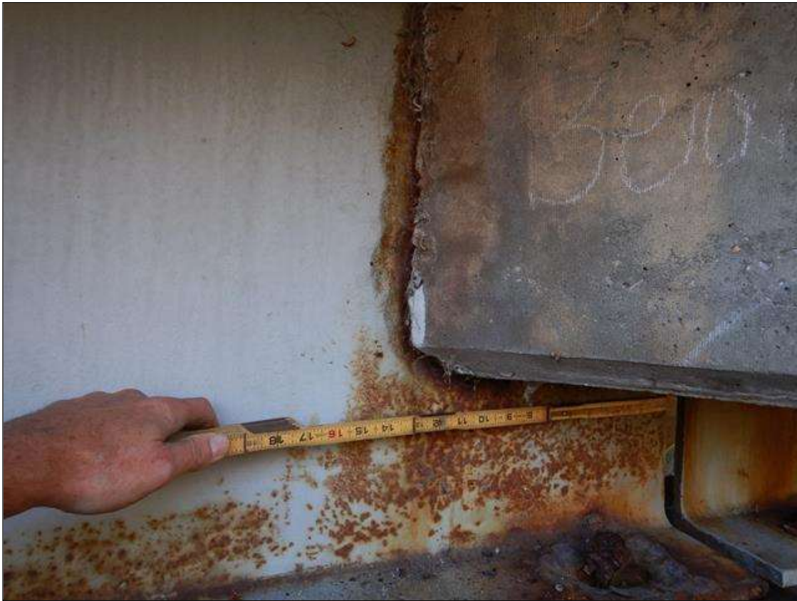
Span 1 Beam 5: [PROMPT ACTION REQUEST] BEAM END AT BENT 1 AT THE INTERFACE WITH THE REINFORCED CONCRETE DIAPHRAGM, THERE IS A BAND OF CORROSION UP TO 2" WIDE WITH SECTION LOSS [AVERAGE 3/16" REMAINS] FOR APPROXIMATELY 1' LONG X UP TO THE FULL HEIGHT OF THE DIAPHRAGM.
