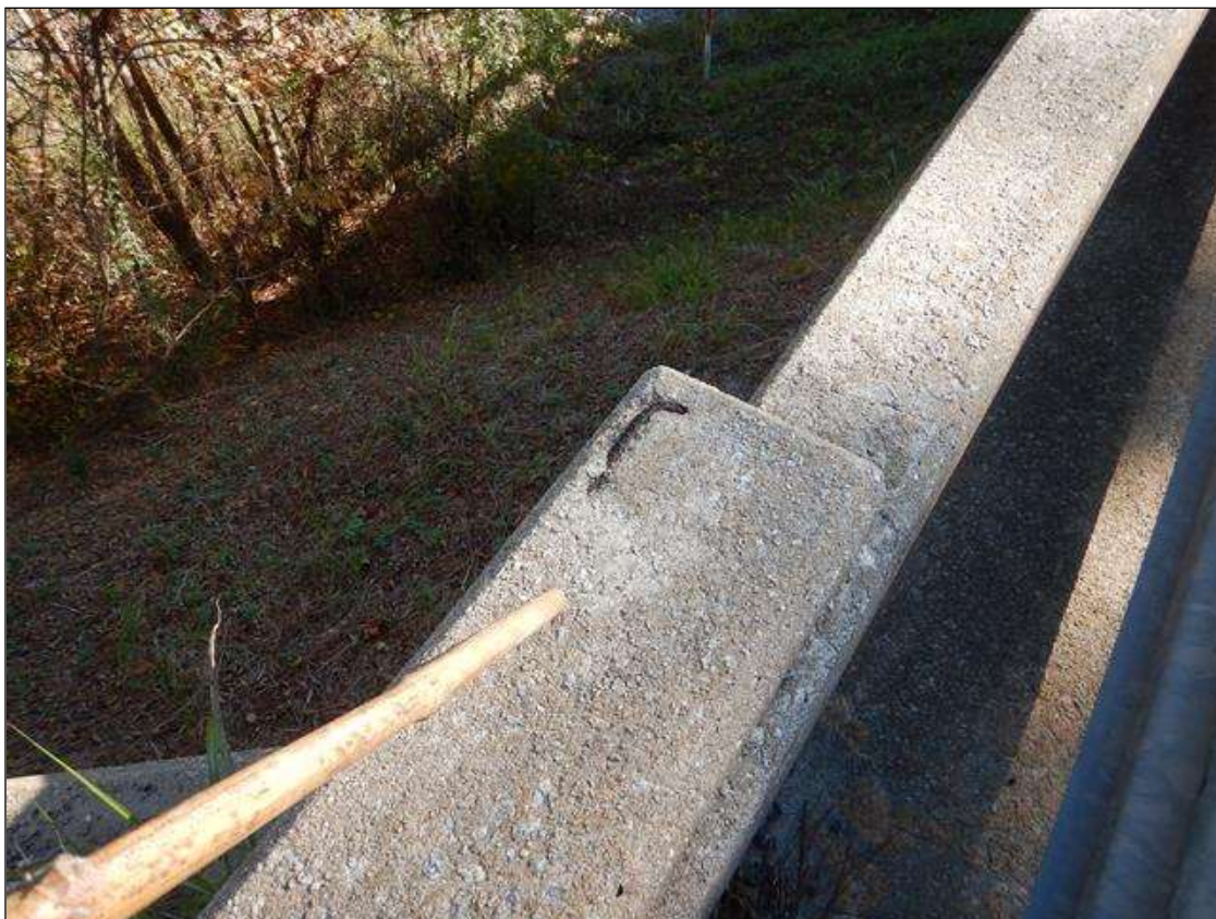
Span 5 Right Bridge Rail: FAR END ON THE TOP OF THE REINFORCED CONCRETE RAIL, EXPOSED REBAR [APPROXIMATELY 5" LONG X 1/2" WIDE] WITH NO MEASURABLE SECTION LOSS
