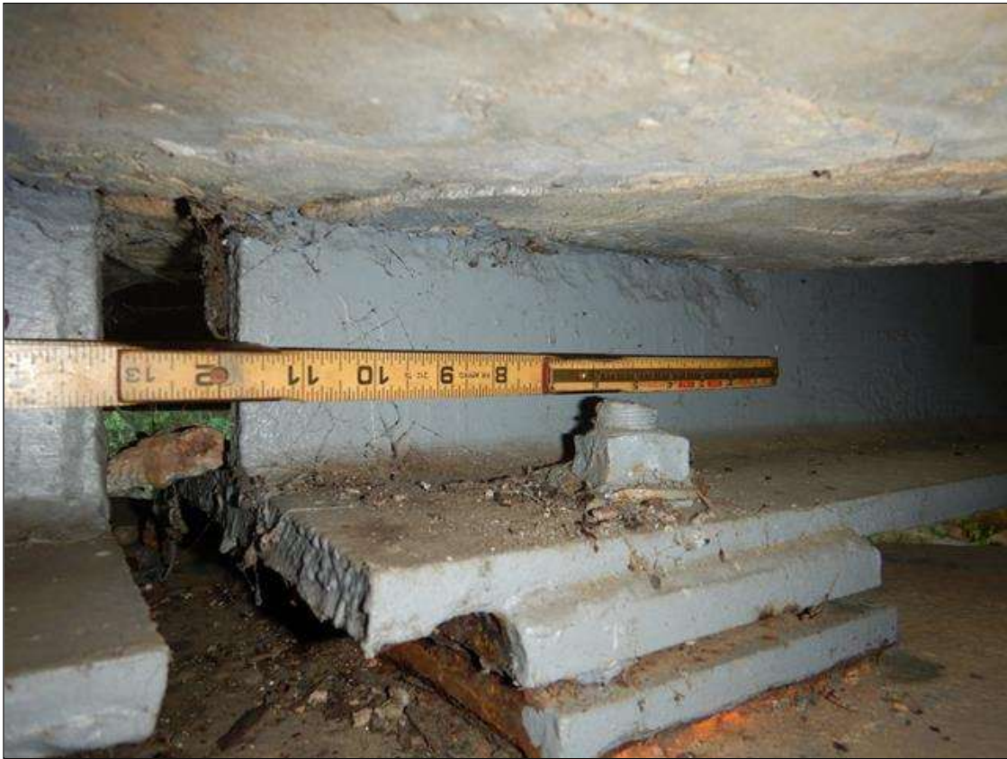
Span 5 Beam 2: PAR--1 FOOT LONG X 2" WIDE AREA OF PREVIOUS CORROSION WITH 1/4" REMAINING SECTION IN WEB AROUND END DIAPHRAGM AT BENT 4 AREA HAS BEEN PAINTED OVER AND ARRESTED.
