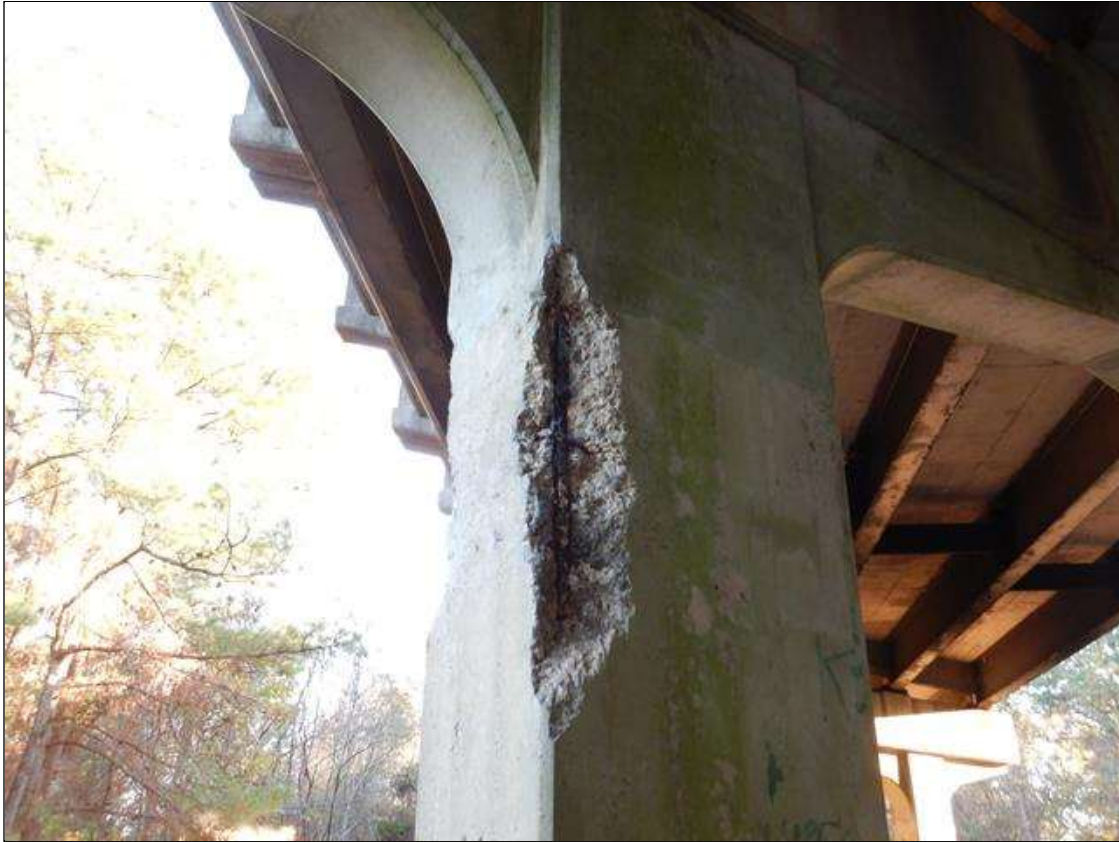
Bent 3 Pile 2: PAR--SPALL WITH EXPOSED REBAR AND BROKEN HORIZONTAL TIE 3 FOOT X 1 FOOT X 4" DEEF IN NORTHEAST CORNER MID HEIGHT WITH SECTION LOSS
