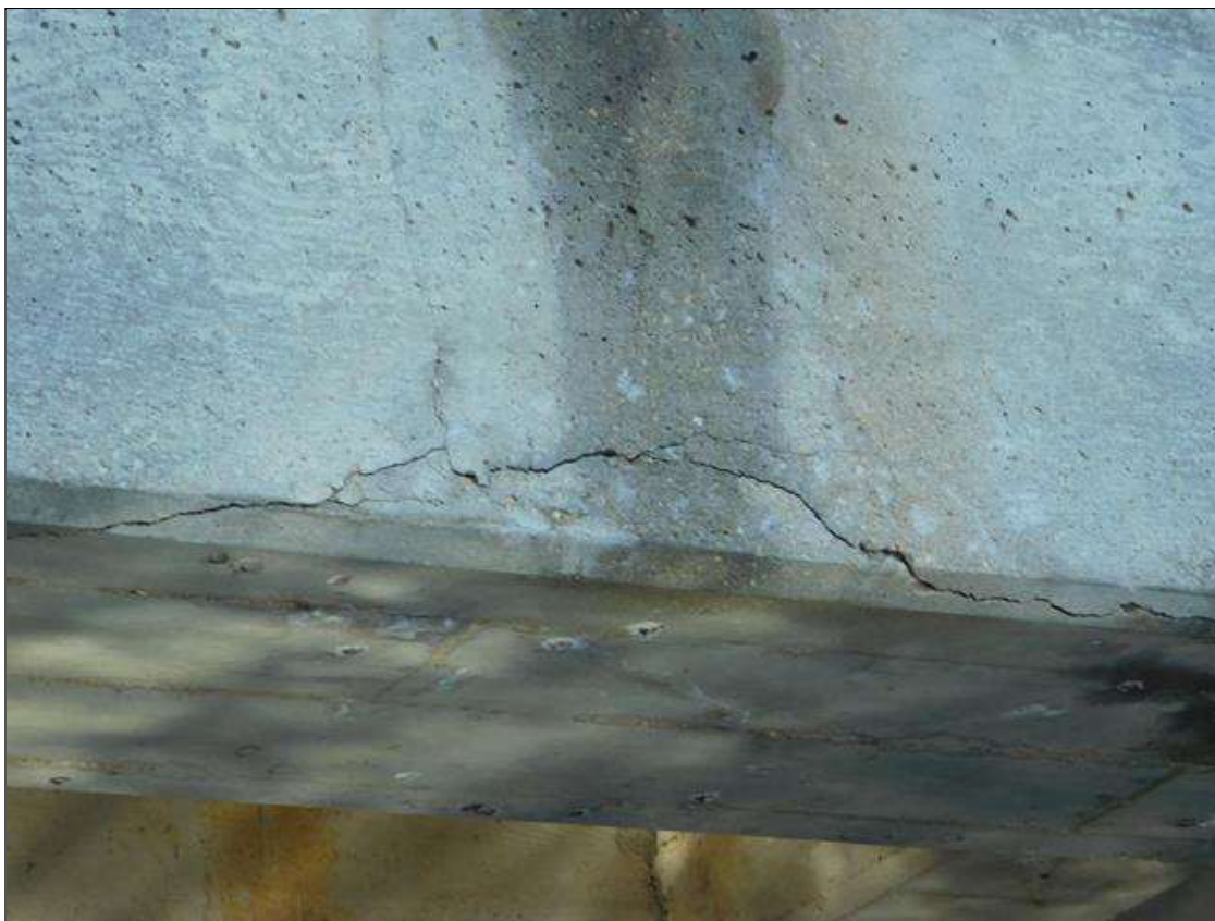
Span 1 Beam 5: CRACKING AND DELAMINATION IN RIGHT SIDE BOTTOM CORNER NEAR MID-SPAN.
