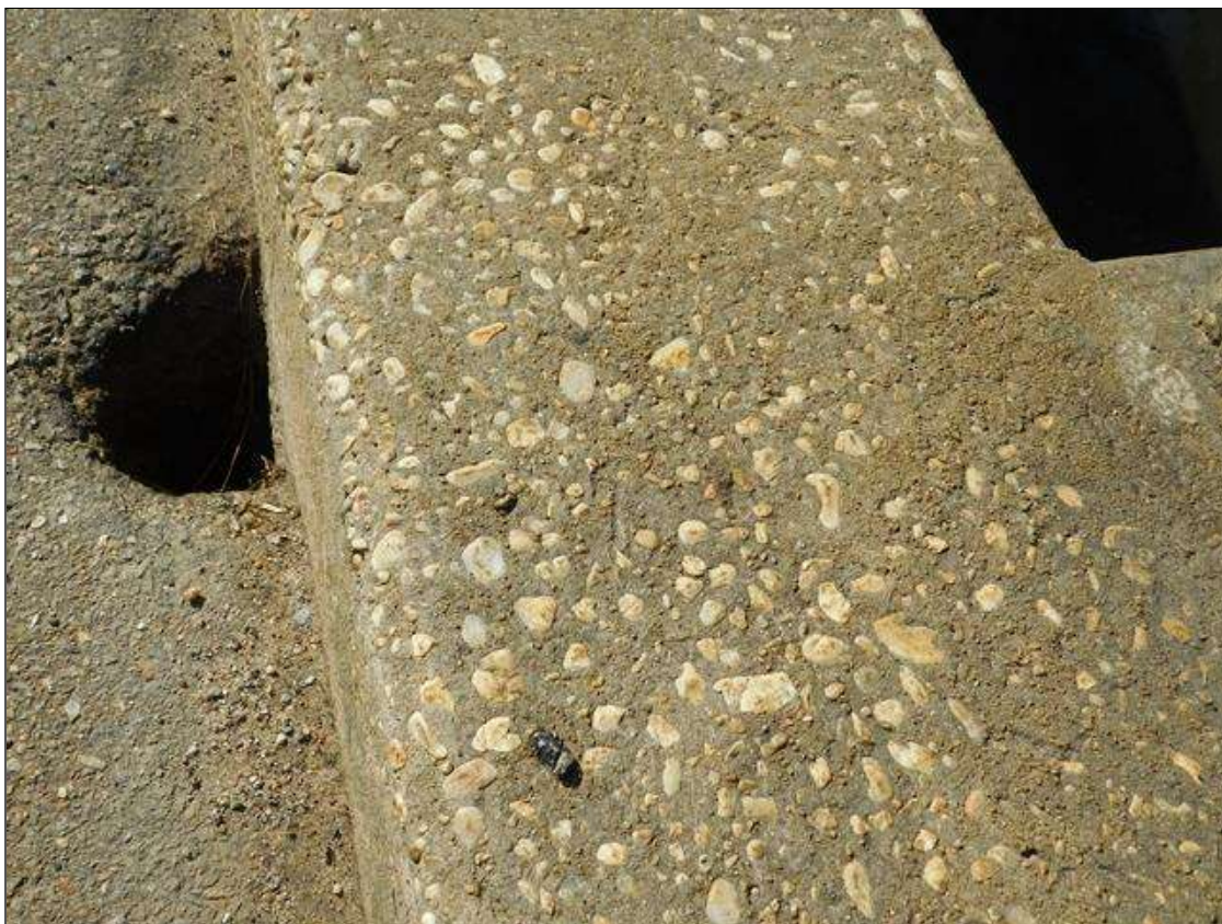
Span 1 Deck: ABRASION ALONG CURBS.
