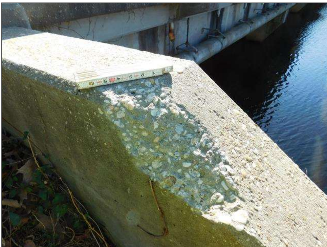
12 IN. LONG X 4 IN. WIDE X 1.25 IN. DEEP SPALL IN LEFT WINGWALL AT END BENT 2.
