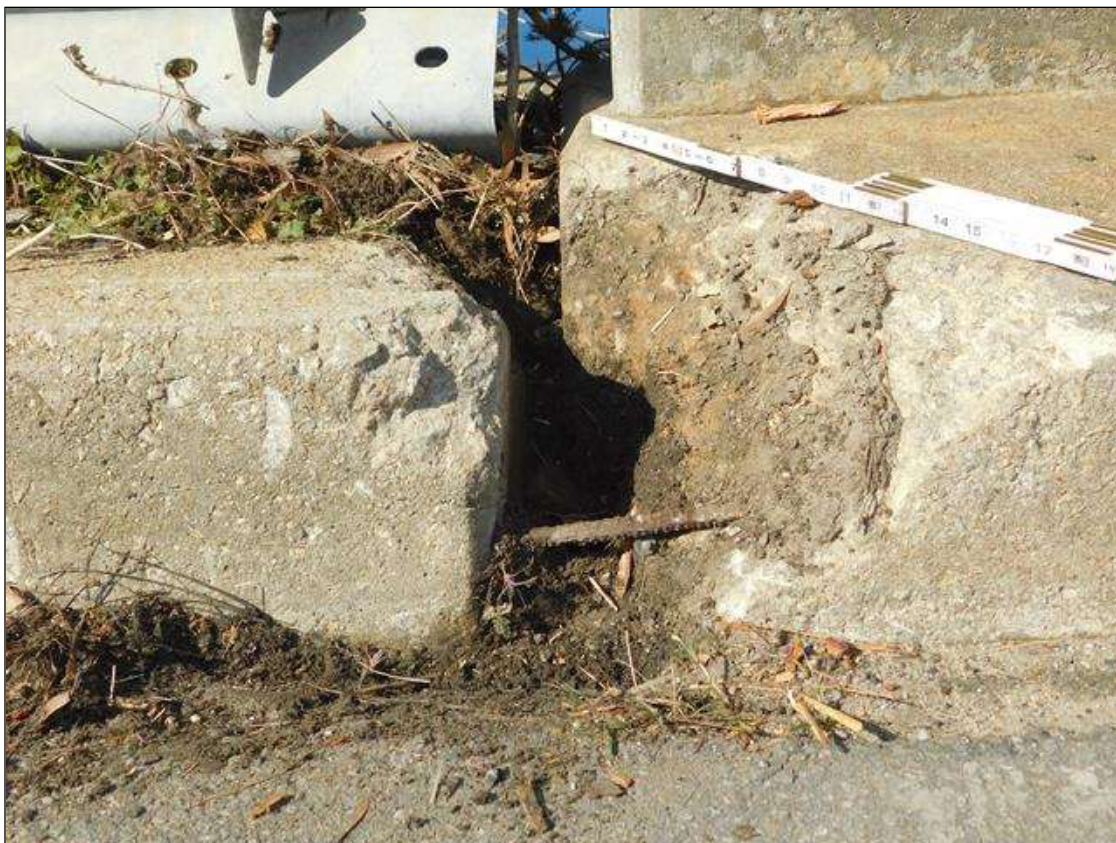
Span 1 Deck: 1 SQUARE FOOT SPALL 8 IN. DEEP WITH EXPOSED REBAR IN LEFT CURB AT END BENT 1.
