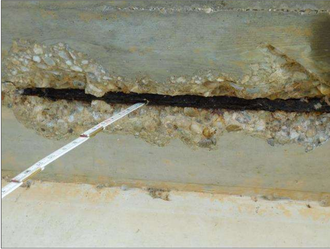
Bent 3 Cap 1: 26" LONG X 7" WIDE X 2" DEEP SPALL WITH SECTION LOSS TO EXPOSED BAR IN BOTTOM OF CAP AT BENT 3 SPAN 3 SIDE UNDER BAY 4 (ESTIMATED 1" DIAMETER BAR REMAINING). PAR ISSUED.
