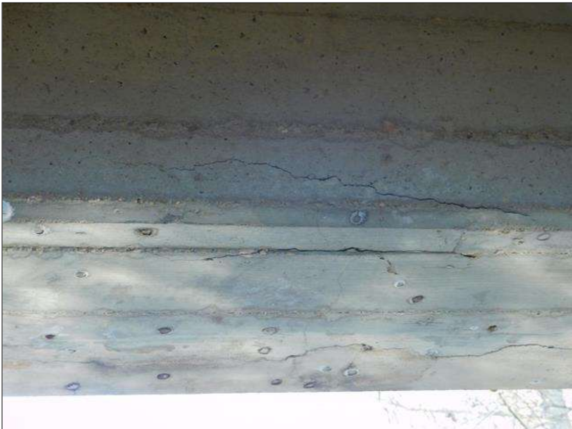
Span 1 Beam 5: LONGITUDINAL CRACKING IN BOTTOM AND LEFT SIDE.
