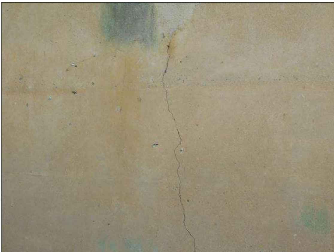
End Bent 1 Abutment: VERTICAL CRACKING 1/16" WIDE IN FACE OF CAP AT GIRDERS 2 & 4 EXTENDING DOWN BREAST WALL.
