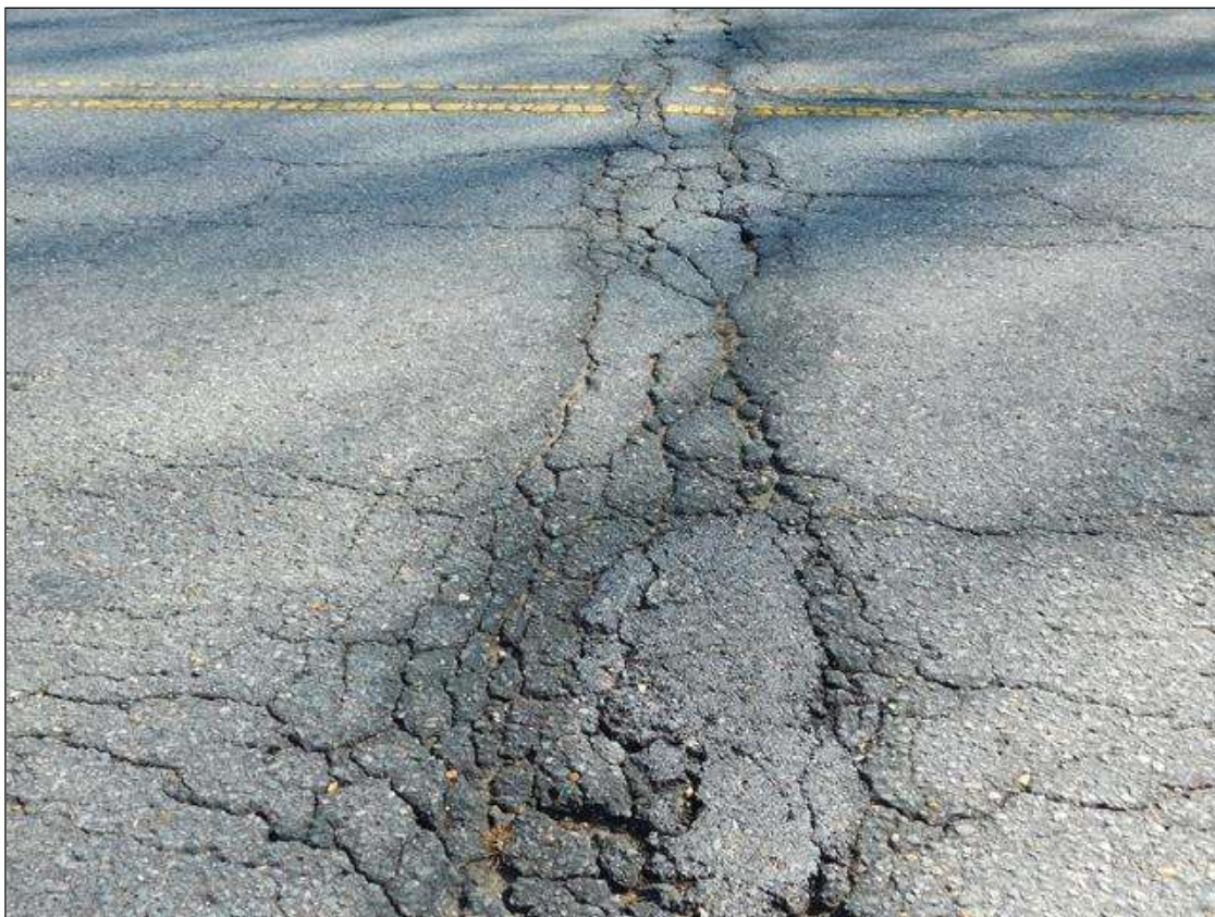
Span 2 Wearing Surface: CRACKING OVER BENT 1.
