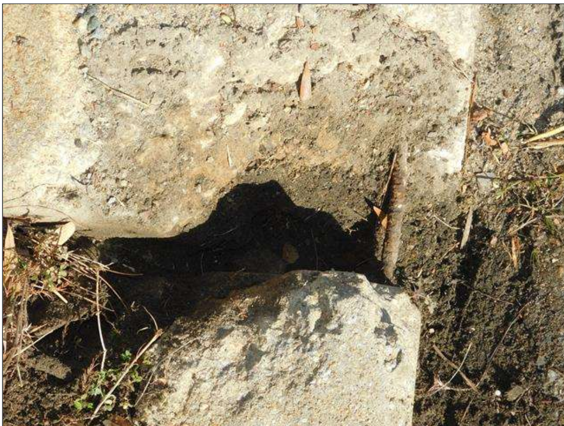
Span 1 Deck: 1 SQUARE FOOT SPALL 8 IN. DEEP WITH EXPOSED REBAR IN LEFT CURB AT END BENT 1.
