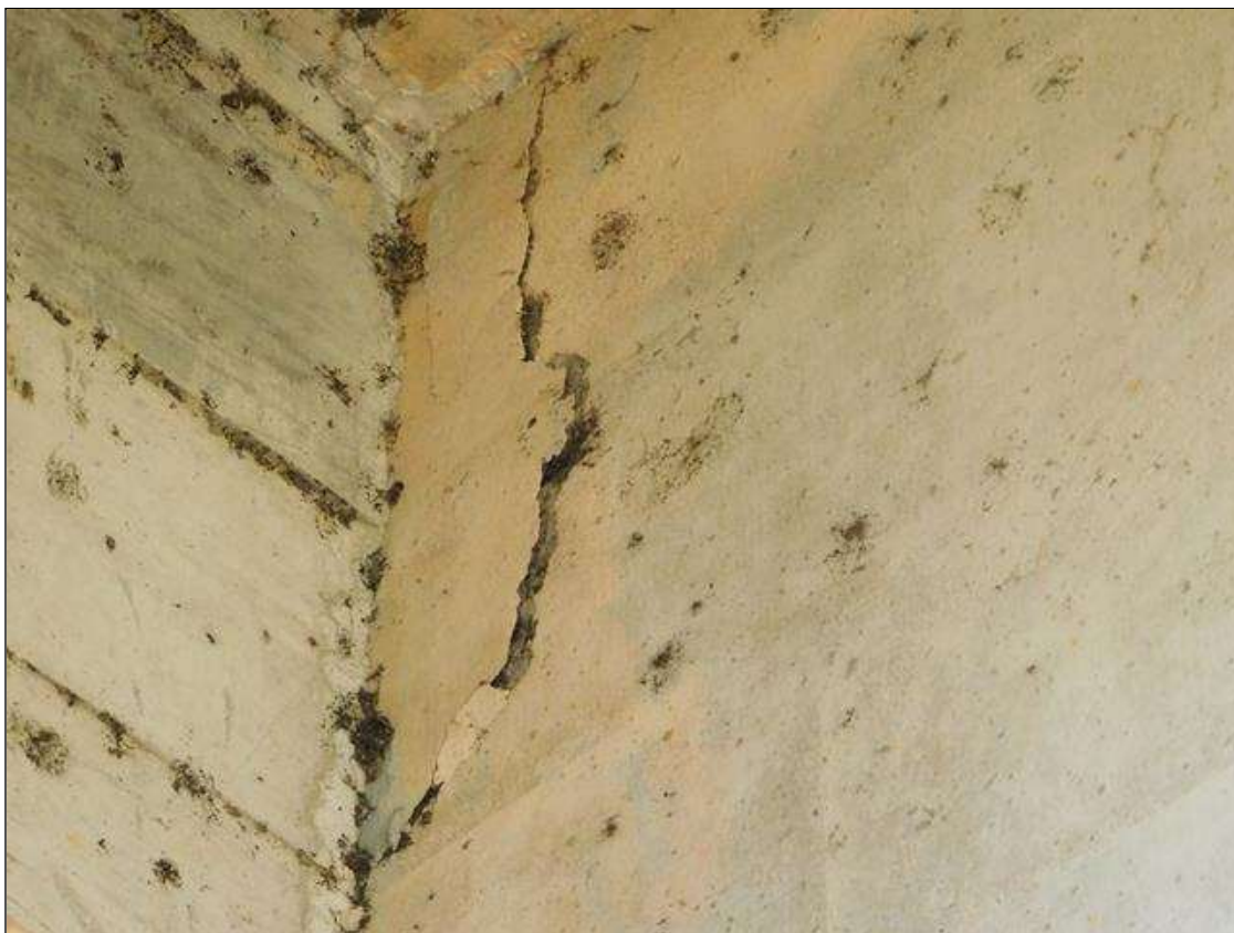
Span 3 Beam 4: DELAMINATION IN RIGHT SIDE WEB AT BENT 3.
