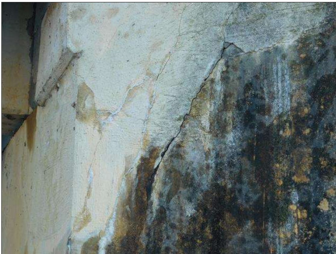
End Bent 1 Abutment: DIAGONAL CRACKING WITH DELAMINATION AND EFFLORESCENCE IN LEFT WINGWALL UNDER GIRDER 1.
