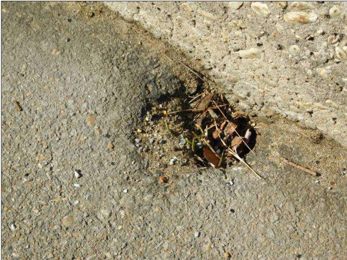
DECK DRAINS BLOCKED BY DECK DEBRIS (SEE DECK DEBRIS)
