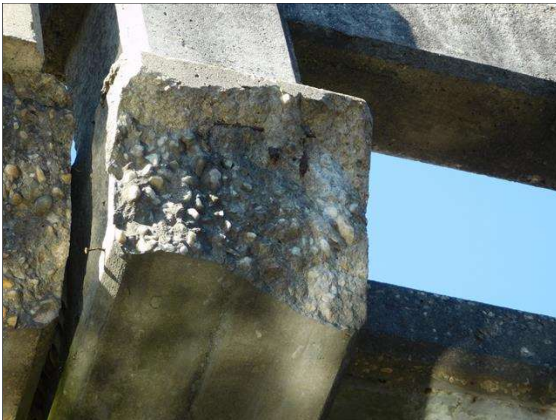
Span 4 Right Bridge Rail: 1 FOOT OF SPALLING 3" DEEP WITH EXPOSED REBAR IN THE GUARDRAIL POST BASE AT BENT 3. PAR ISSUED.
