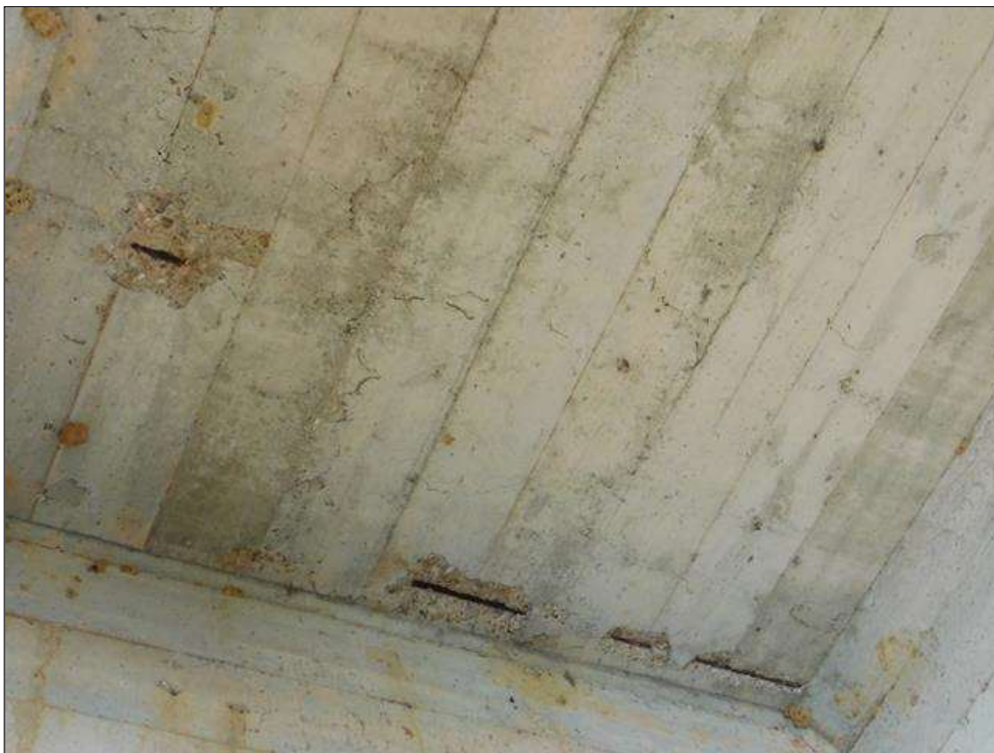
Span 1 Deck: 3 SQUARE FOOT OF SHALLOW SPALLING WITH EXPOSED REBAR IN BOTTOM OF DECK BAY 3 AT END BENT 1.
