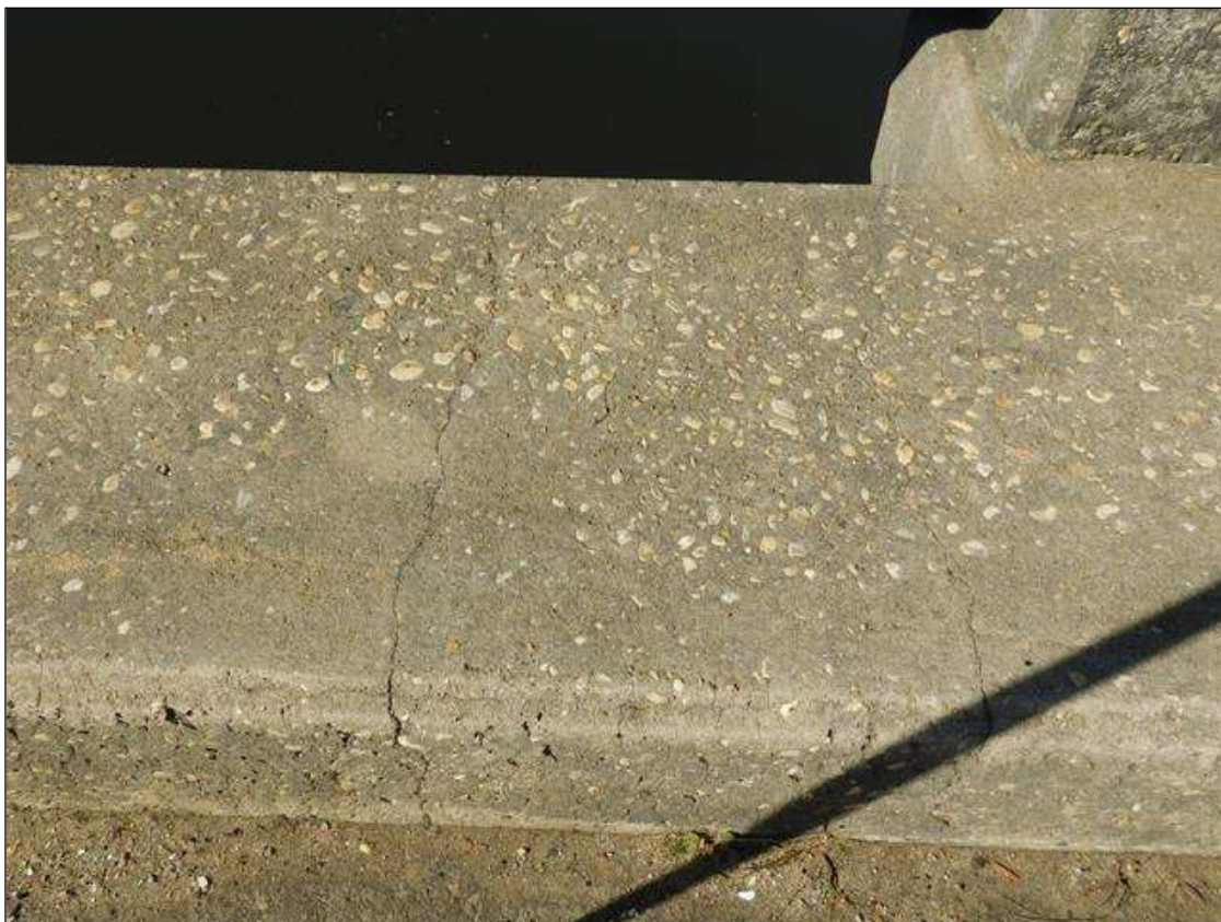
Span 1 Deck: CRACKING IN CURBS.
