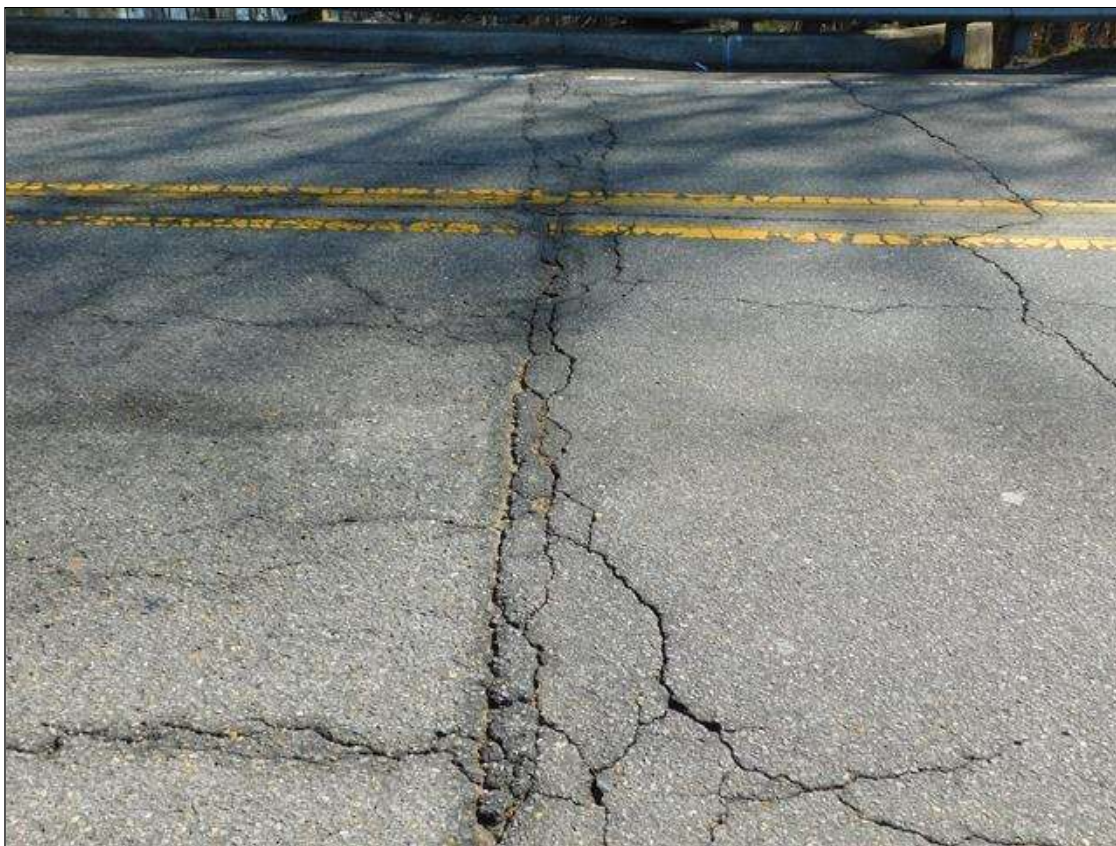
Span 1 Wearing Surface: 28 SQUARE FEET OF CRACKING NEAR END BENT 1.
