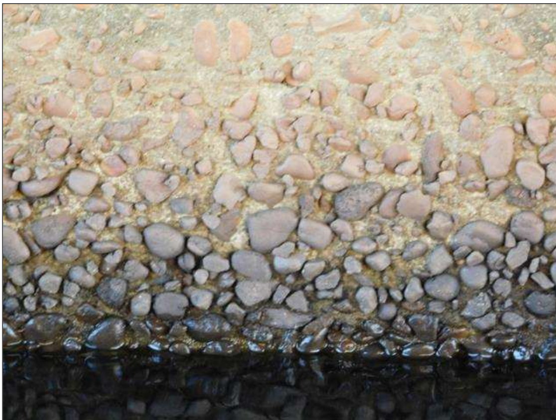
Bent 1 Pile 1: ABRASION WITH COARSE AGGREGATE EXPOSED FROM WATERLINE UP 3 FEET.
