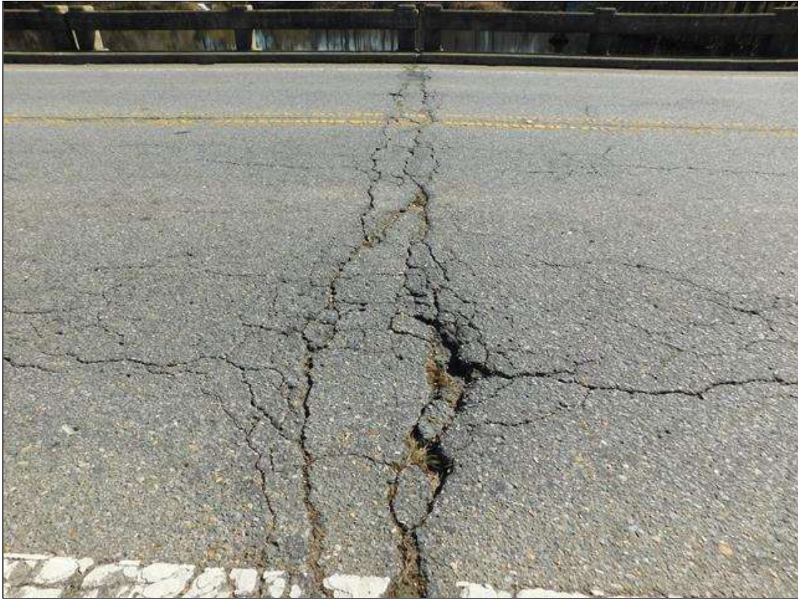
Span 3 Wearing Surface: CRACKING OVER BENT 2.
