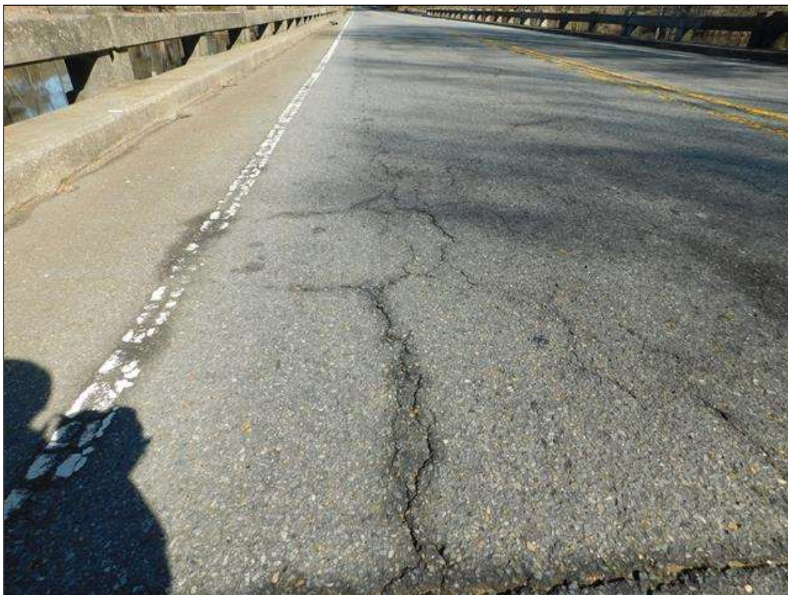
Span 1 Wearing Surface: CRACKING ALONG TRAVEL LANES.
