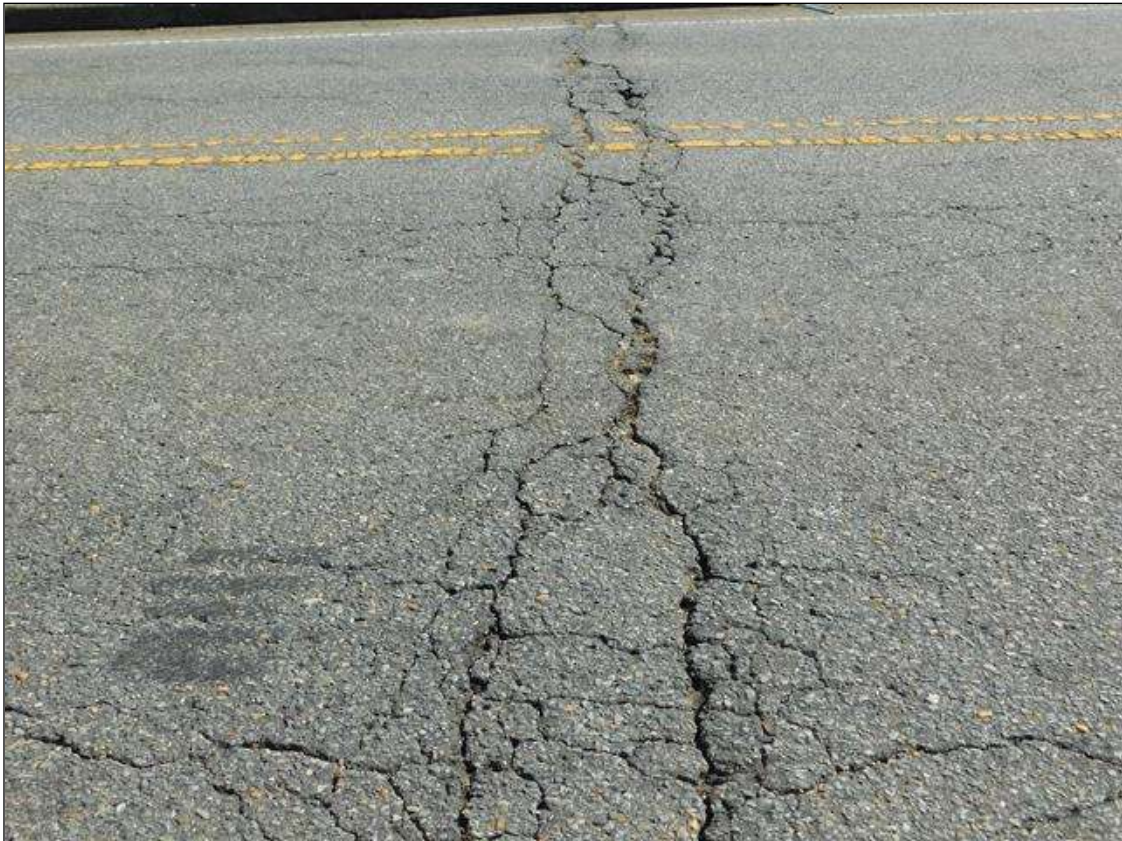
Span 4 Wearing Surface: CRACKING OVER BENT 3 AND END BENT 2 AND ALONG TRAVEL LANES.
