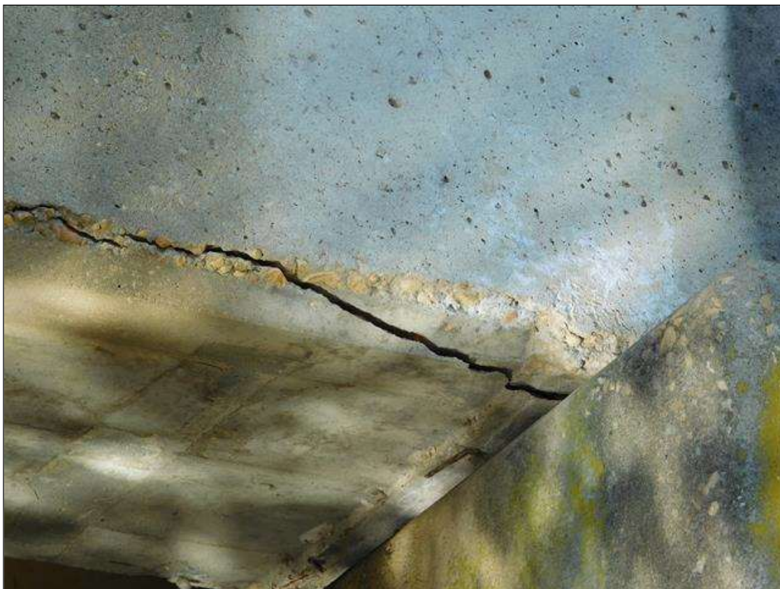
Span 3 Beam 5: 3/16" WIDE LONGITUDINAL CRACK 2' LONG IN BOTTOM RIGHT CORNER AT BENT 3.
