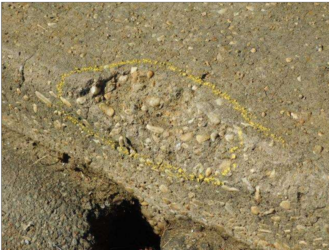
Span 1 Deck: SPALL IN THE LEFT CURB AT BENT 1.
