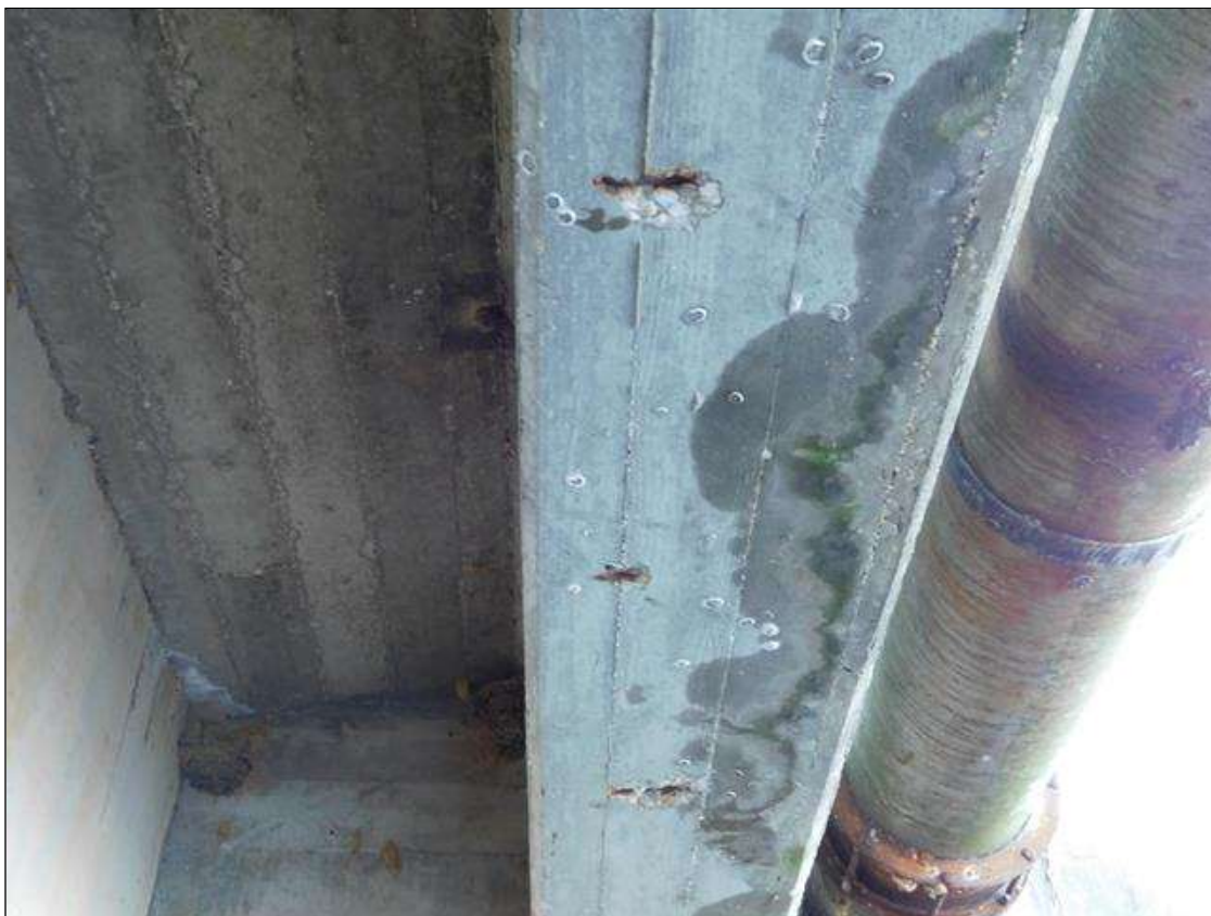
Span 1 Beam 1: SHALLOW SPALLS WITH EXPOSED REBAR IN BOTTOM OF GIRDER UP TO 6 FT. OUT FROM END BENT 1.
