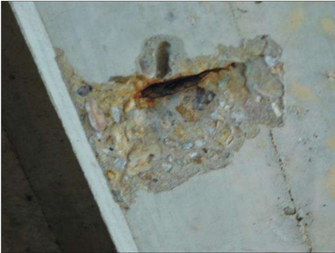
Span 1 Beam 4: 6" DIAMETER SPALL 3/4" DEEP WITH EXPOSED STEEL.
