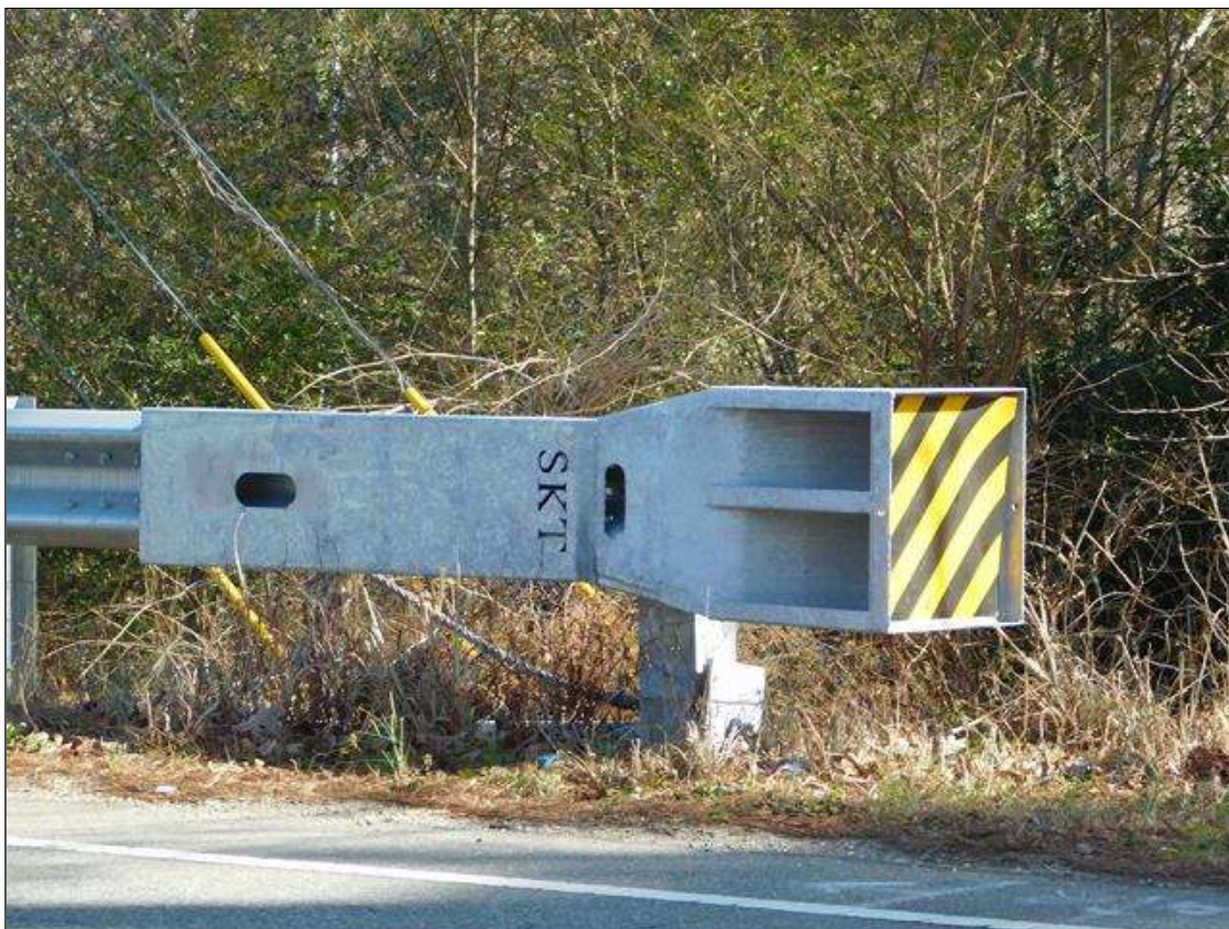
APPROACH GUARDRAIL TERMINAL END RIGHT SIDE AT SOUTH END
