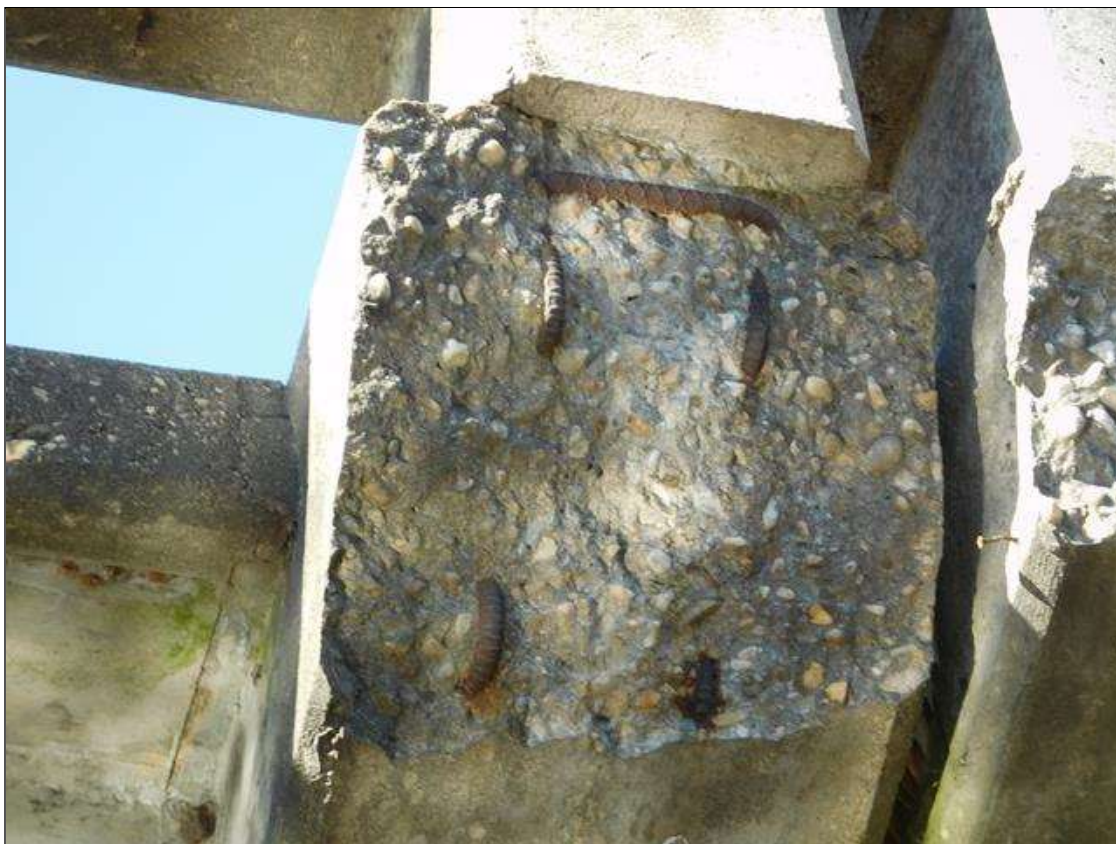
Span 3 Right Bridge Rail: 1 FOOT OF SPALLING 3" DEEP WITH EXPOSED REBAR IN THE GUARDRAIL POST BASE AT BENT 3. PAR ISSUED.
