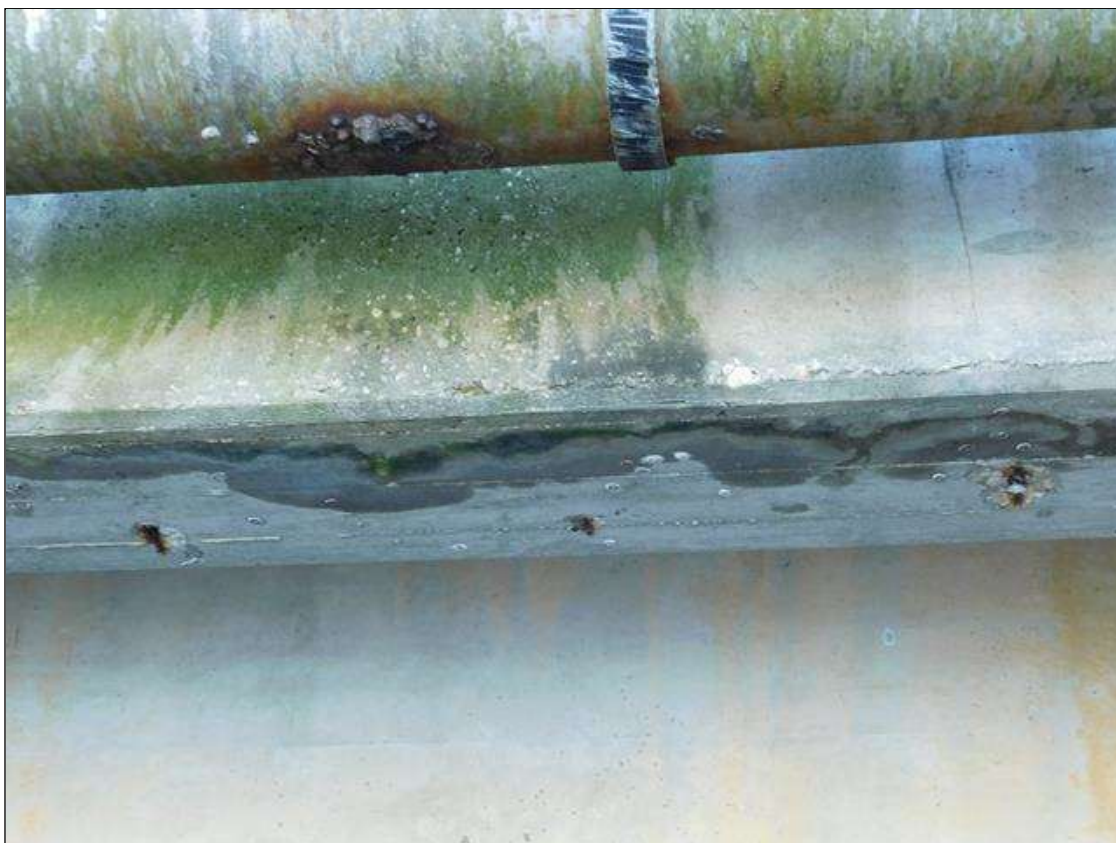
Span 1 Beam 1: SHALLOW SPALLS WITH EXPOSED REBAR IN BOTTOM OF GIRDER UP TO 6 FT. OUT FROM END BENT 1.
