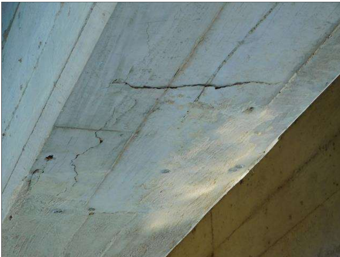
Span 1 Beam 4: 12" DIAMETER DELAMINATION IN BOTTOM OF BEAM AT MID-SPAN.
