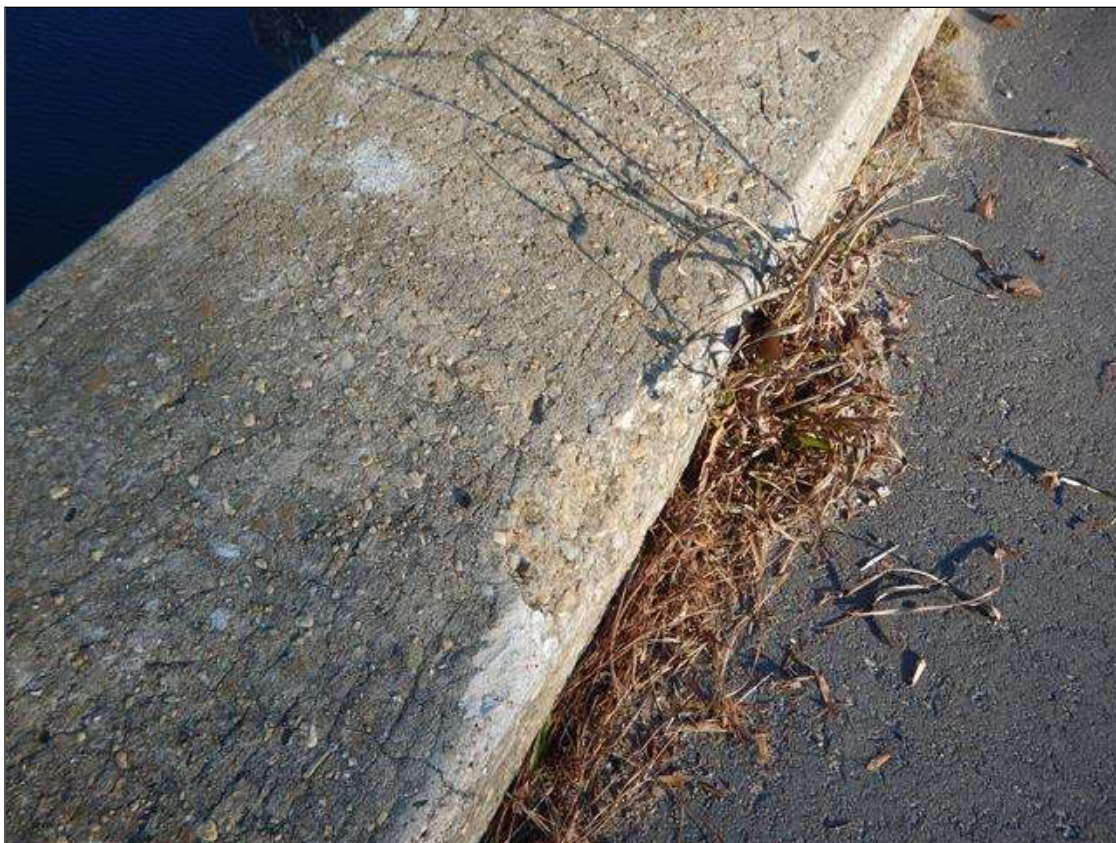
Span 1 Left Bridge Rail: 6 INCHES LONG X 3 INCHES WIDE X 1 INCH DEEP AT 2 FEET FROM BENT 1
