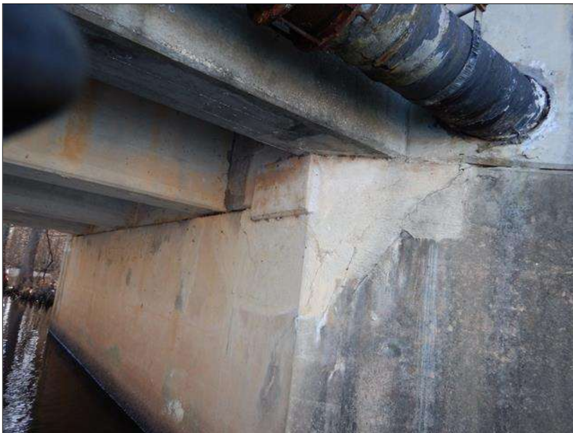
End Bent 1 Abutment: SOUND PATCHING IN CAP UNDER GIRDERS 1, 2 & 3.
