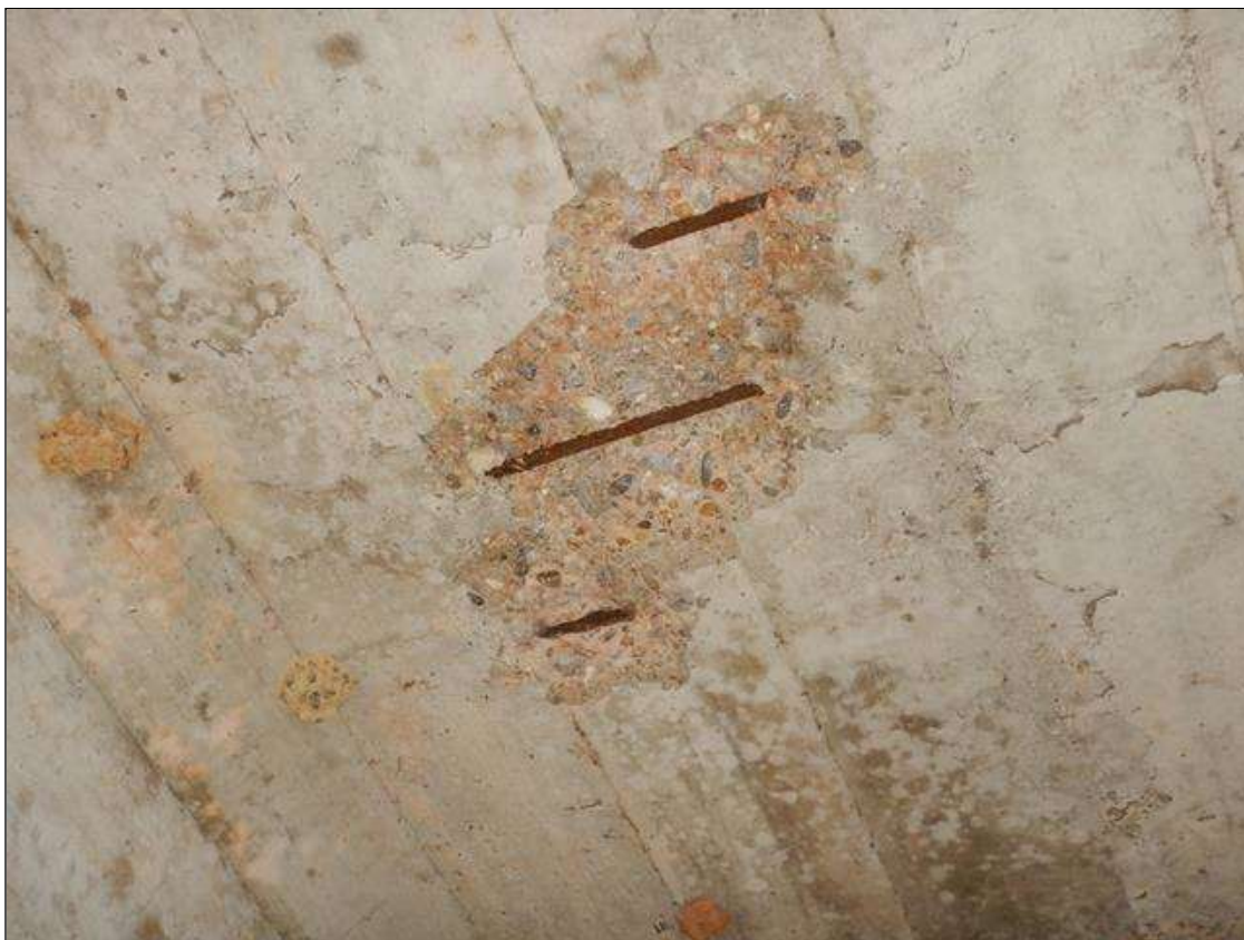
Span 1 Deck: 8 INCHES WIDE X 18 INCHES LONG X 1/2 INCHES DEEP SPALL WITH EXPOSED REBAR IN BOTTOM OF THE DECK AT BAY 3 NEAR END BENT 1 ADJACENT BEAM 4.
