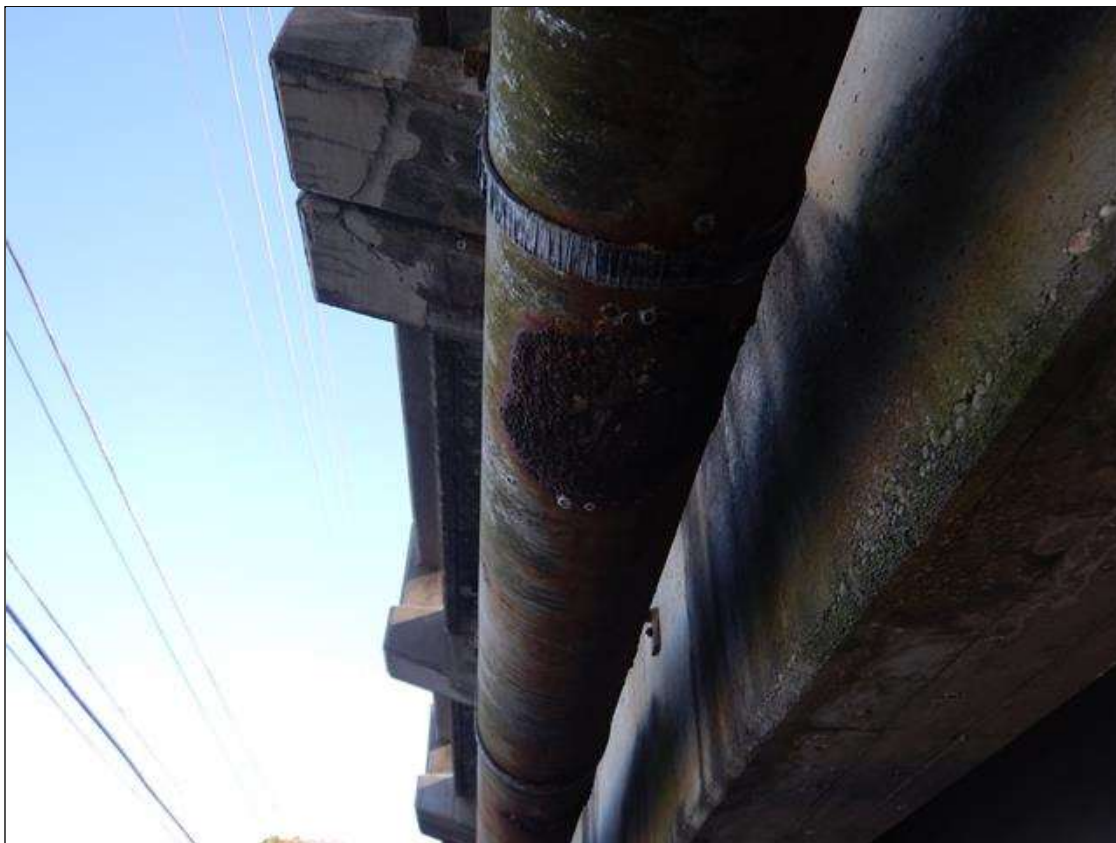
AREAS OF CORROSION ALONG BOTTOM OF 12 INCHES UTILITY PIPE ALONG THE LEFT OVERHANG
