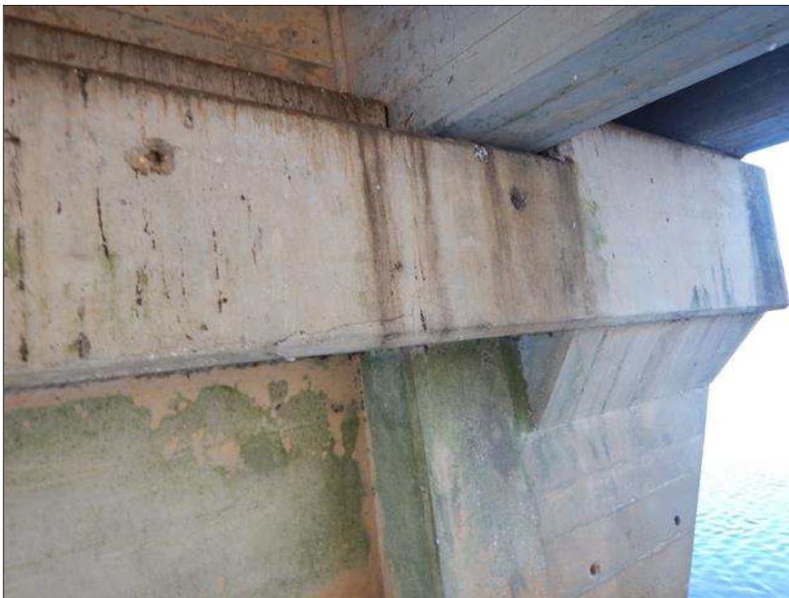
Bent 2 Cap 1: CRACKING ALONG THE BOTTOM CORNER OF CAP FOR 2 FEET LONG X 1- 1/2 INCHES HIGH UNDER BEAM 4
