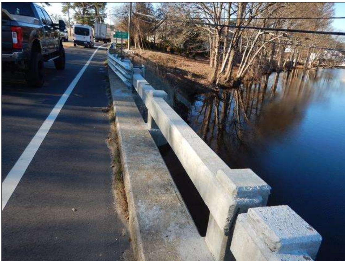
30 FEET LEFT RAIL IN SPAN 1 BEGINNING AT END BENT 1 HAS BEEN REPAIRED
