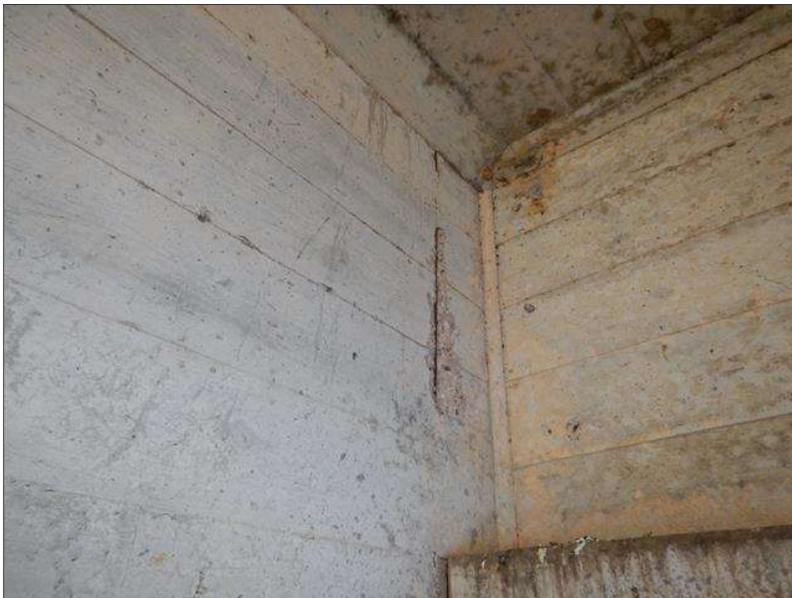
Span 3 Beam 3: 14 INCHES HIGH X 6 INCHES WIDE SPALL WITH EXPOSED STEEL IN THE LEFT SIDE AT BENT 2.
