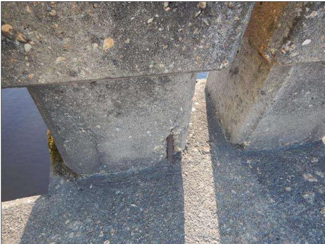
Span 2 Right Bridge Rail: 1 FEET OF EXPOSED REBAR WITH SPALL AT POST 4 FROM BENT 1
