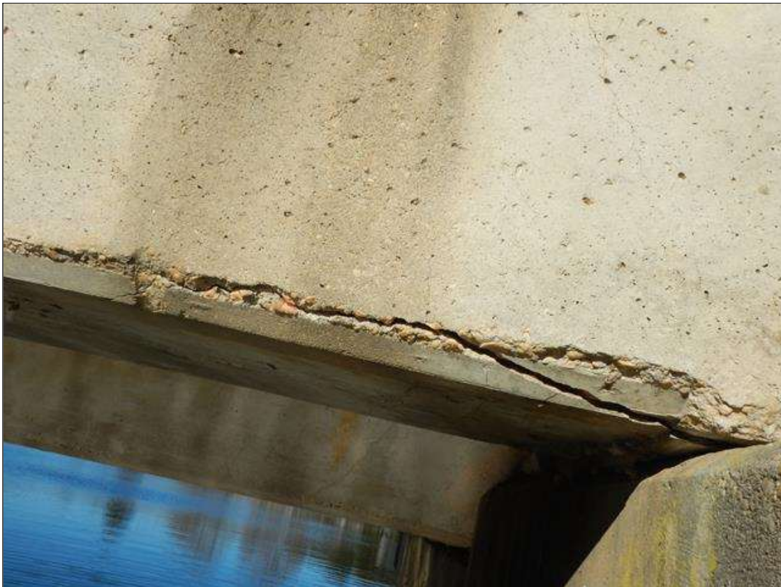
Span 3 Beam 5: 3/16 INCHES WIDE LONGITUDINAL CRACK 2 FEET LONG IN BOTTOM RIGHT AND LEFT CORNER AT BENT 3.
