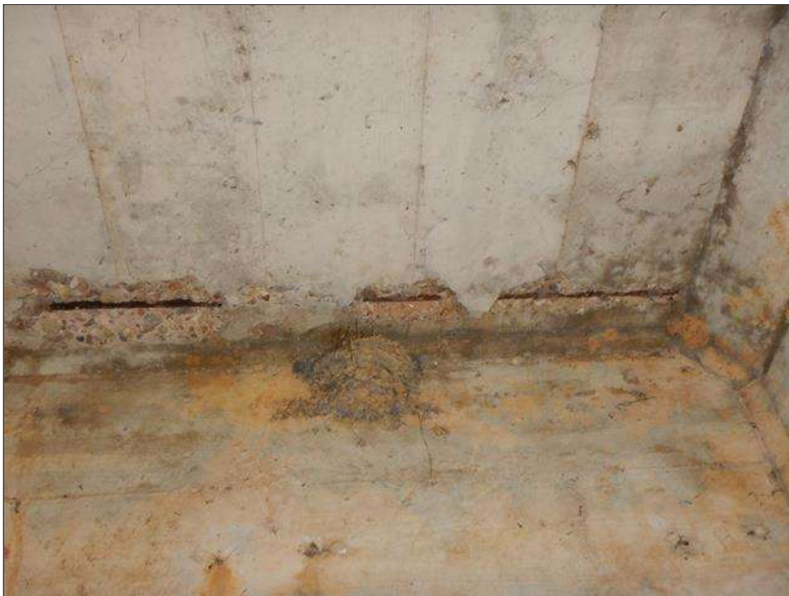
Span 1 Deck: 3 FEET WIDE X 5 INCHES LONG X 1/2 INCH DEEP SPALL WITH EXPOSED REBAR IN THE BOTTOM OF THE DECK BAY 3 AT END BENT 1
