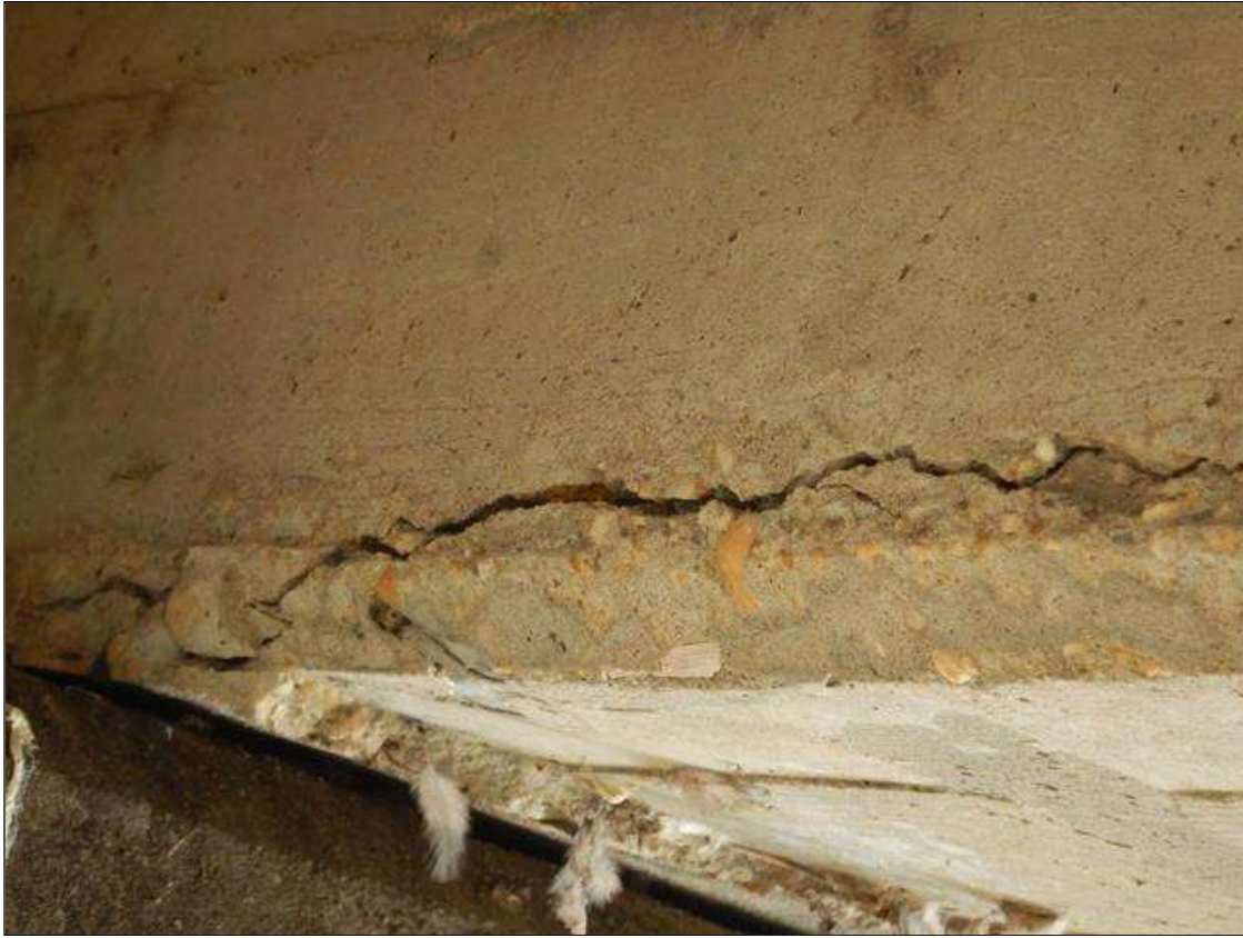
Span 3 Beam 5: 3/16 INCHES WIDE LONGITUDINAL CRACK 2 FEET ALONG IN BOTTOM RIGHT AND LEFT CORNER AT BENT 3.
