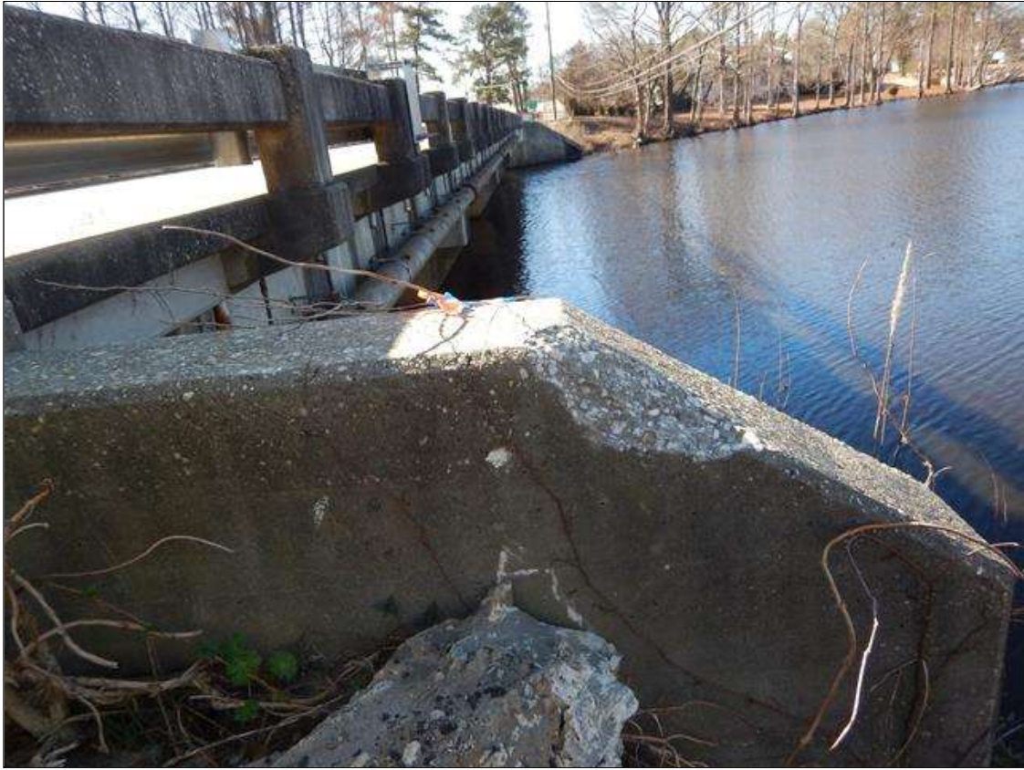
1 FOOT LONG X 6 INCHES WIDE X 1.5 INCHES DEEP SPALL TOP OF LEFT WINGWALL AT END BENT 2
