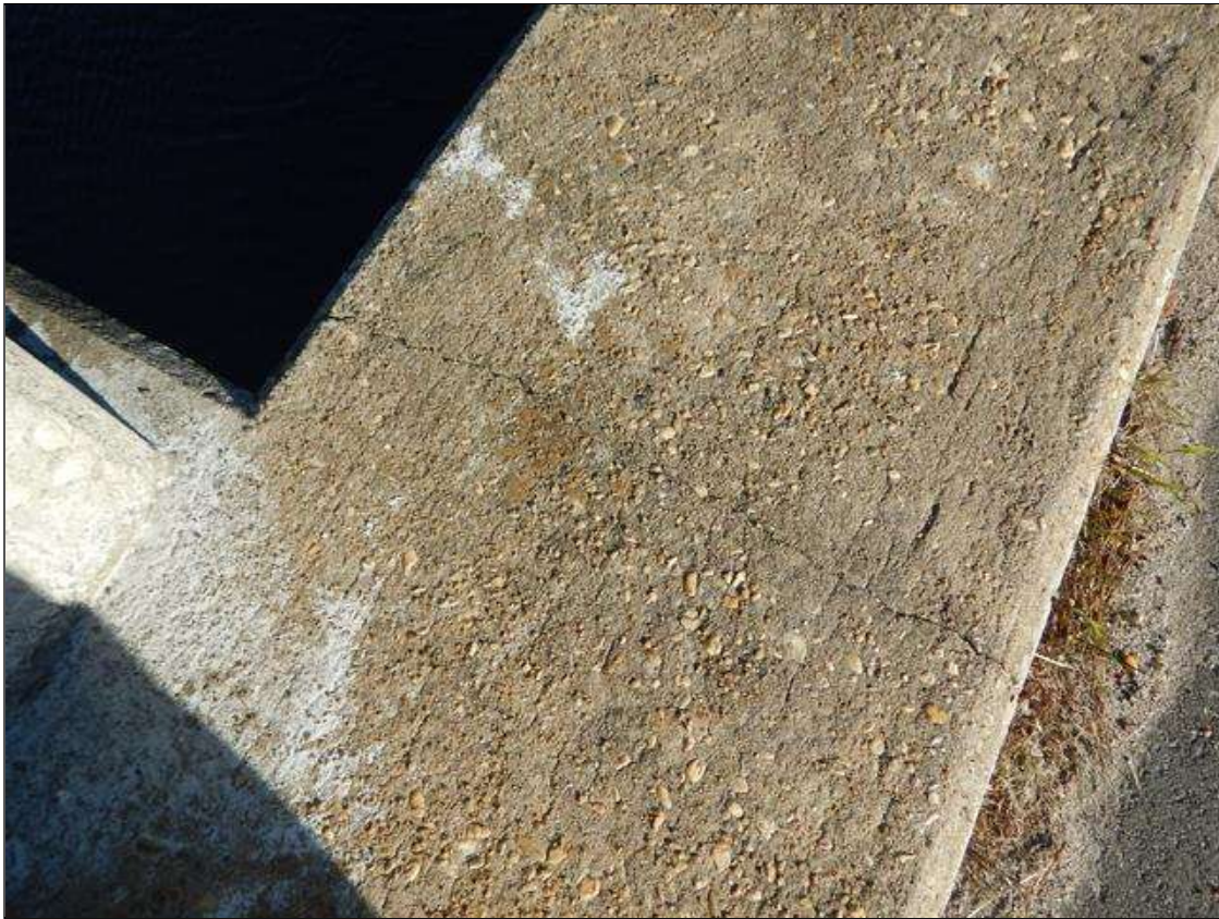
Span 2 Left Bridge Rail: TRANSVERSE CRACK 8 FEET FROM BENT 2
