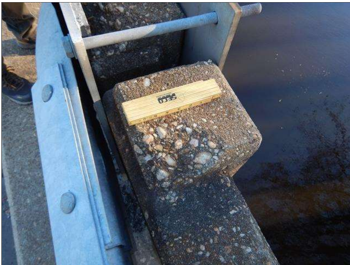
Span 1 Right Bridge Rail: 6 INCHES WIDE X 3 INCHES LONG X 1/2 INCH DEEP OF SPALLING/DELAMINATION POST 3 .
