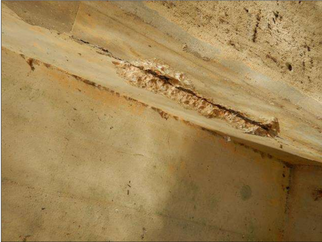
Bent 3 Cap 1: (PAR) 26 INCHES LONG X 7 INCHES WIDE X 2 INCHES DEEP SPALL WITH SECTION LOSS TO EXPOSED BAR IN BOTTOM OF CAP AT BENT 3 SPAN 3 SIDE UNDER BAY 4 (ESTIMATED 1 INCH DIAMETER BAR REMAINING).
