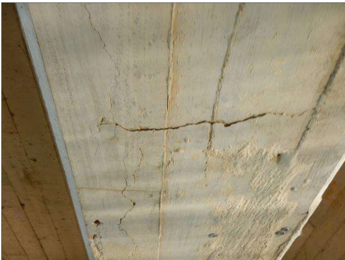
Span 1 Beam 4: 12 INCHES DIAMETER DELAMINATION IN BOTTOM OF BEAM AT MID-SPAN.
