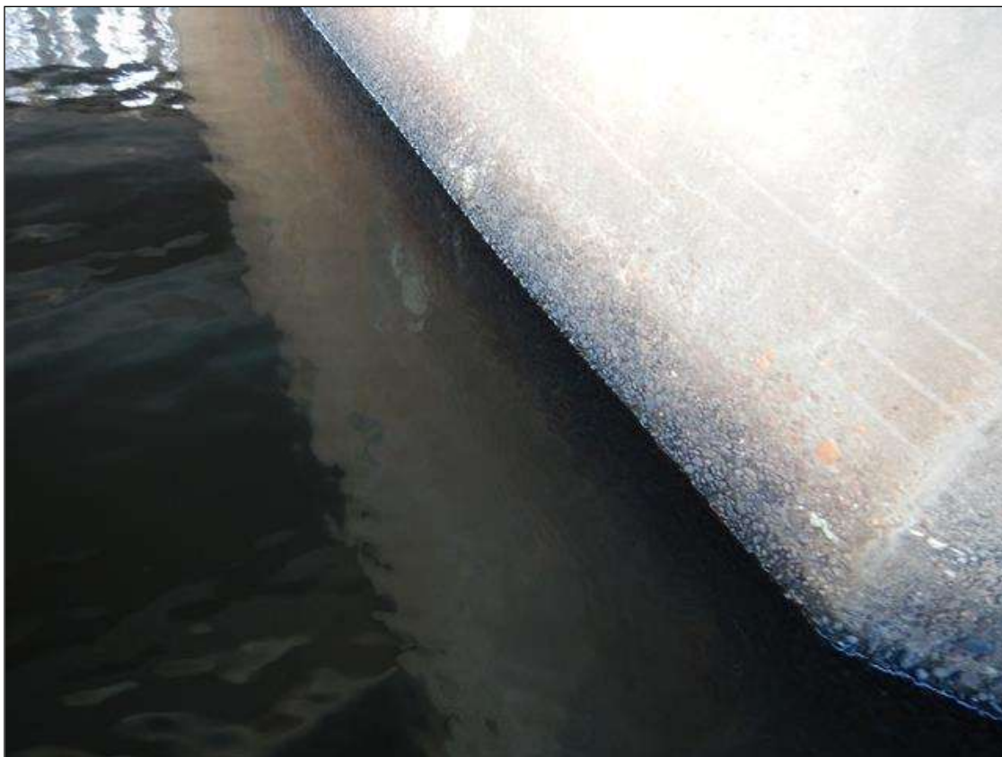
End Bent 1 Abutment: 57 FEET OF ABRASION WITH COARSE AGGREGATE EXPOSED FROM WATERLINE UP 3 FEET
