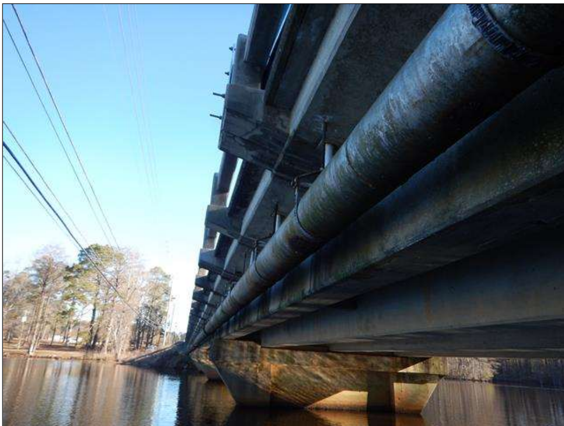
UTILITY UNDER LEFT OVERHANG
