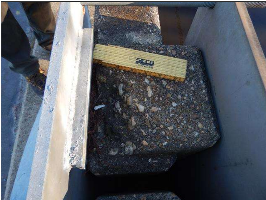
Span 1 Right Bridge Rail: 7 INCHES LONG X 3 INCHES WIDE X 2 INCHES DEEP WITH EXPOSED REBAR AT POST 4.
