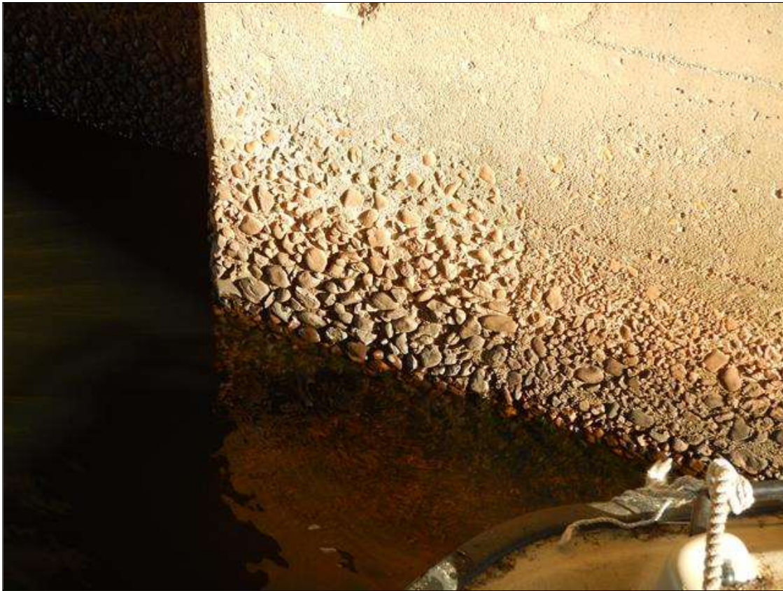
Bent 1 Pile 1: ABRASION WITH COARSE AGGREGATE EXPOSED FROM WATERLINE UP 3 FEET. ALSO NOTE FRONT OF BOAT.
