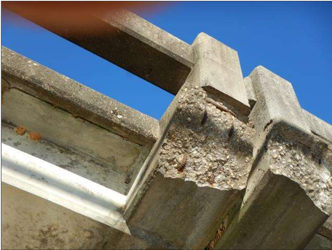
Span 3 Right Bridge Rail: (PAR) 1 FOOT OF SPALLING 3 INCHES DEEP WITH EXPOSED REBAR IN THE GUARDRAIL POST BASE AT BENT 3.
