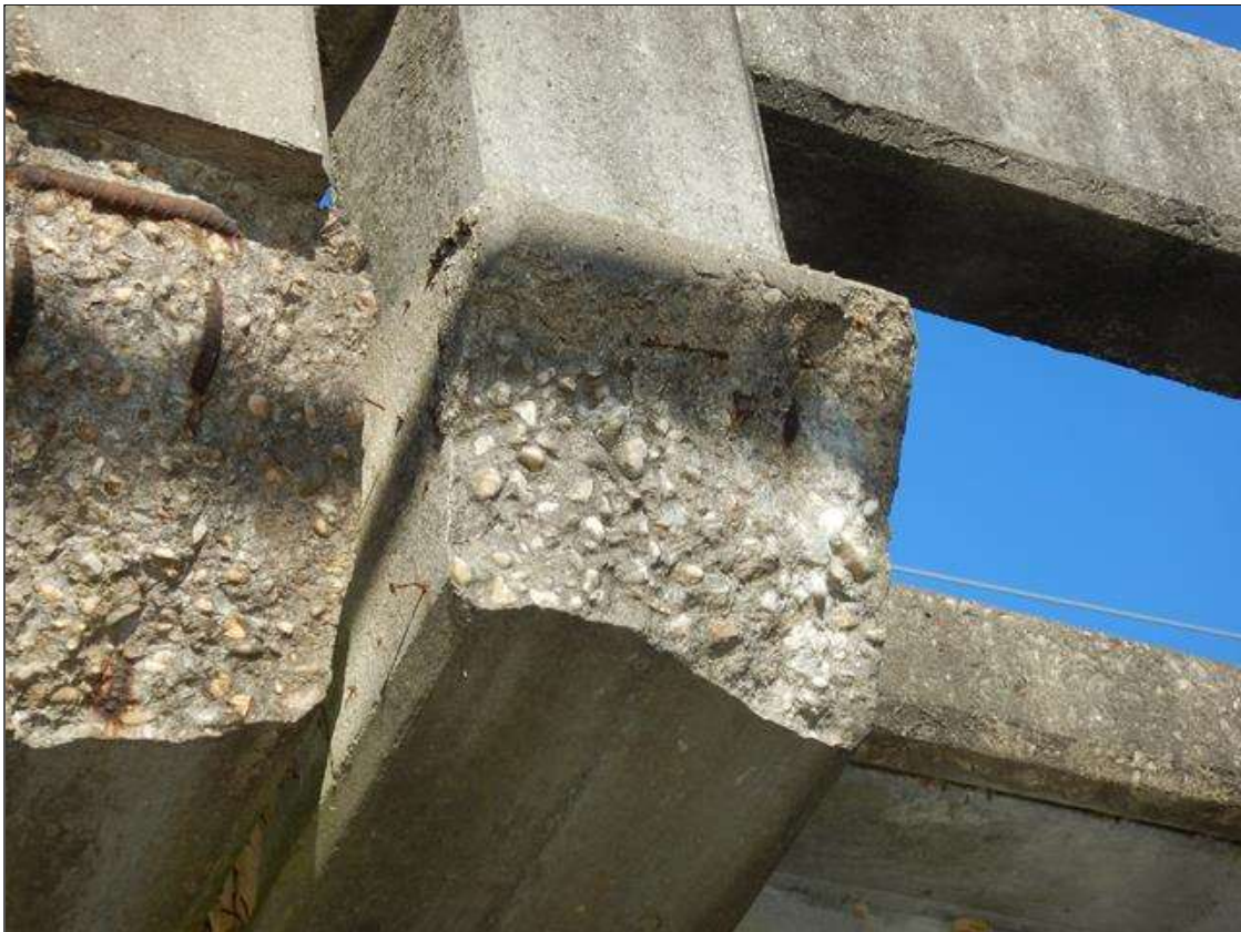
Span 4 Right Bridge Rail: (PAR) 1 FOOT OF SPALLING 3 INCHES DEEP WITH EXPOSED REBAR IN THE GUARDRAIL POST BASE AT BENT 3.
