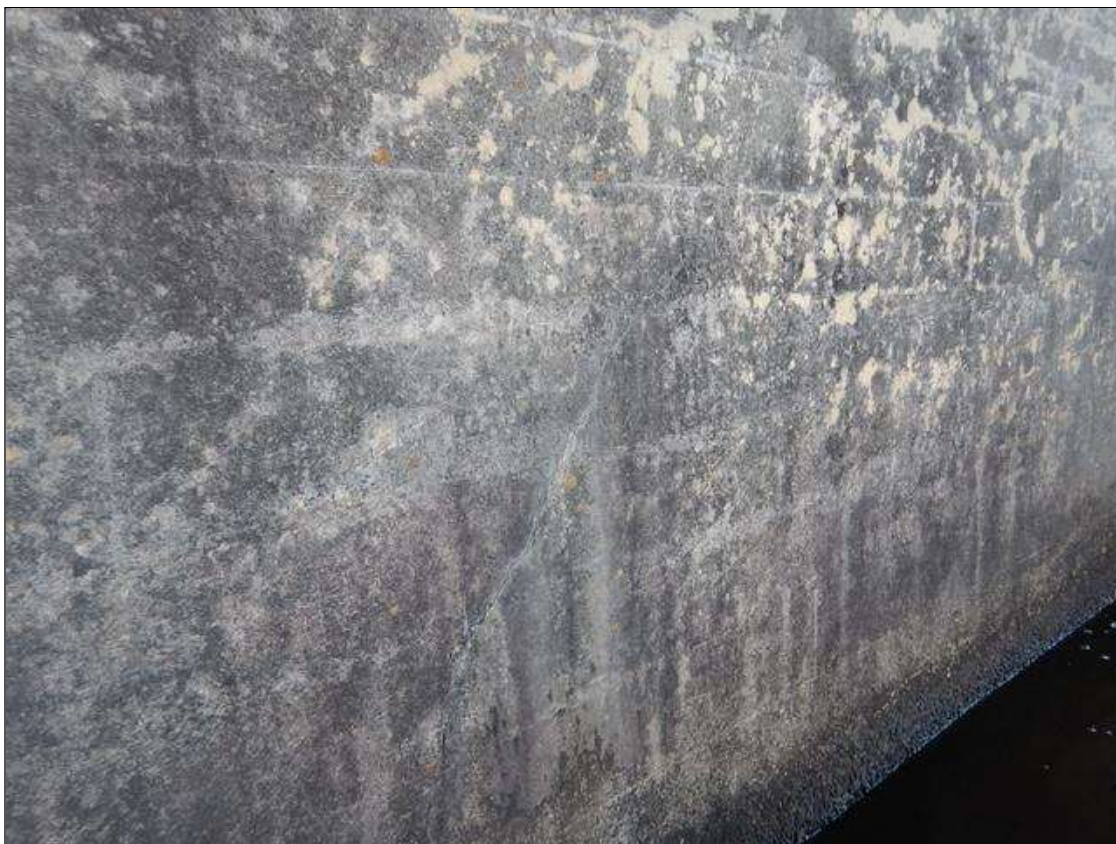
End Bent 1 Abutment: VERTICAL DIAGONAL CRACK 8 FEET LONG IN SOUTH WEST WINGWALL
