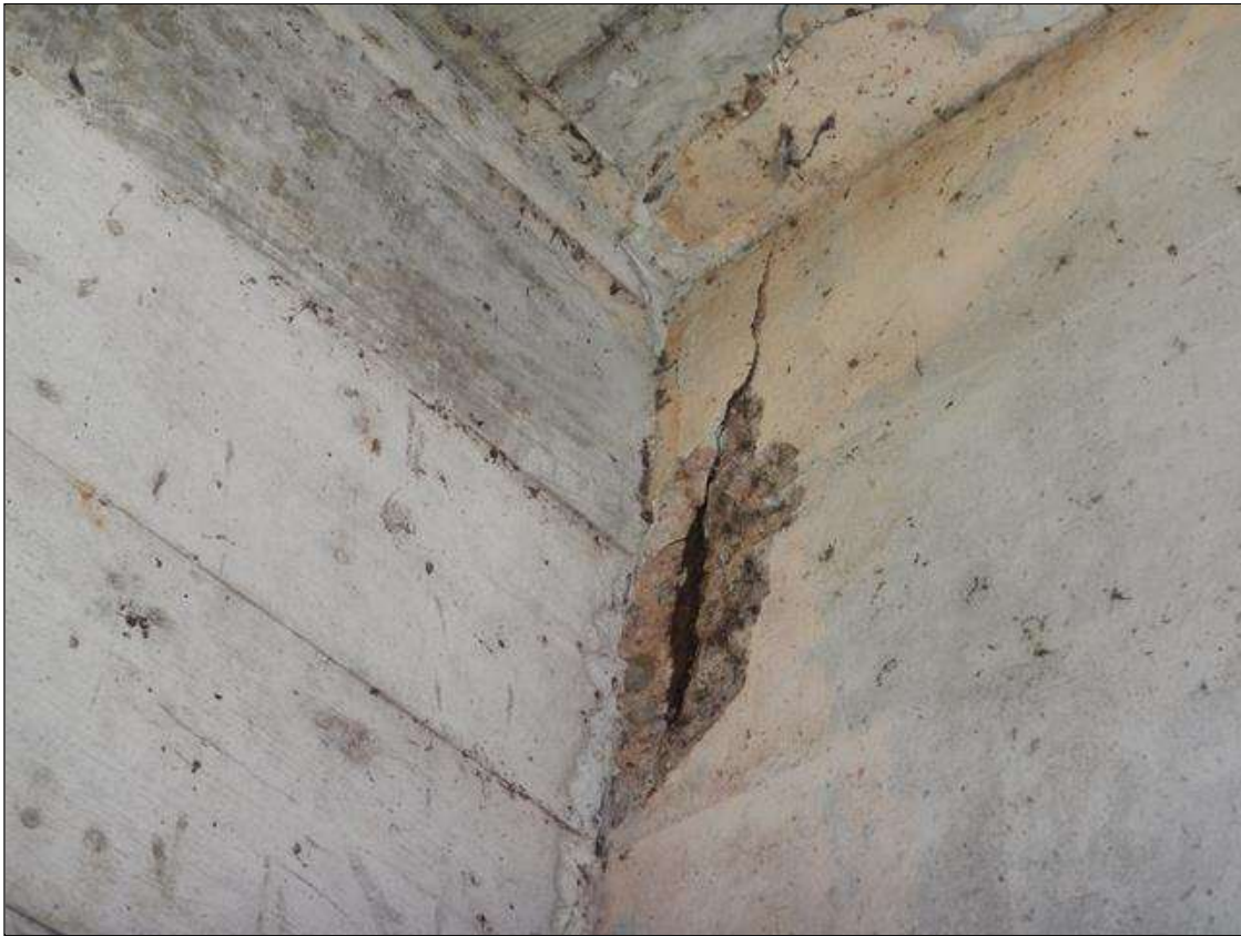
Span 3 Beam 4: 18 INCHES HIGH X 4 INCHES WIDE X 3/4 INCHES DEEP SPALL WITH EXPOSED REBAR IN RIGHT SIDE WEB AT BENT 3.
