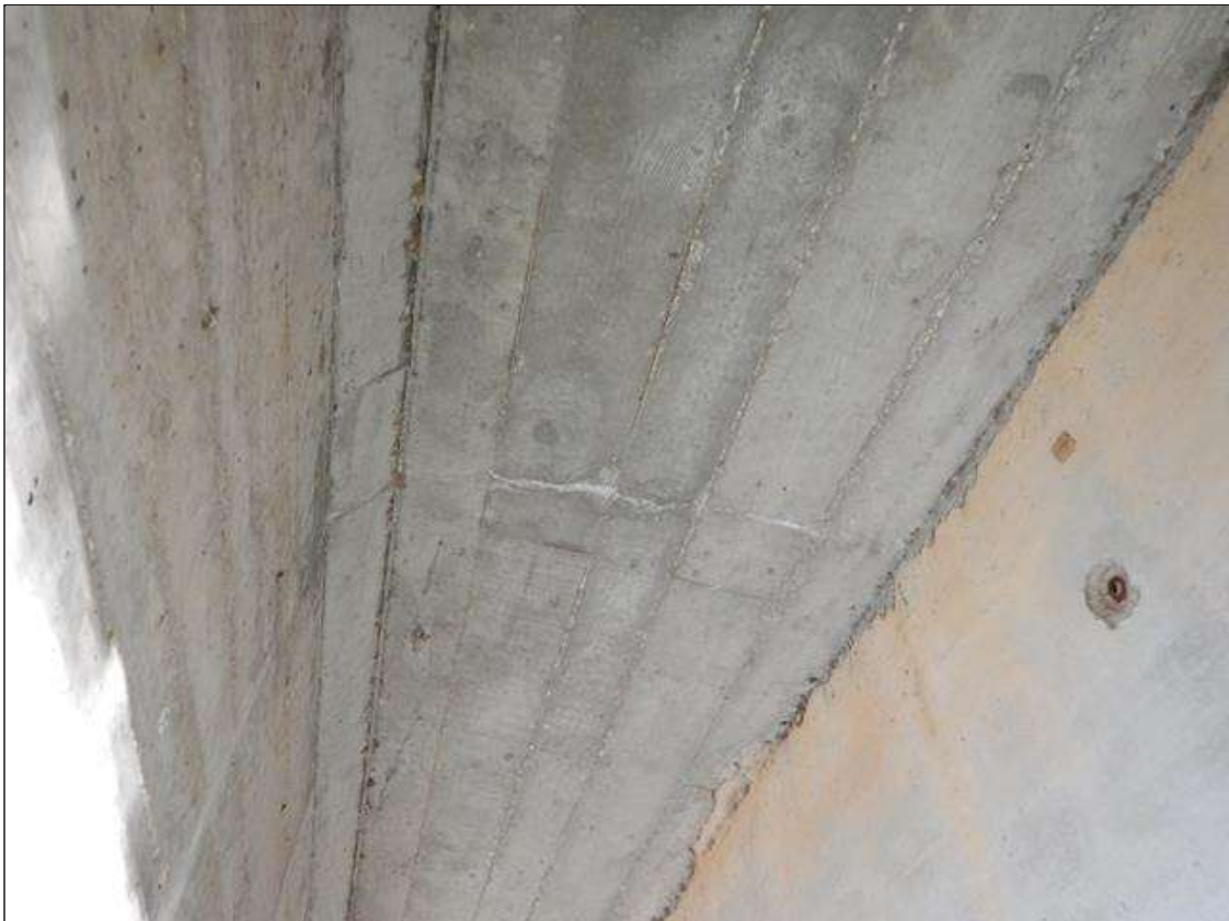
Span 2 Deck: SCATTERED TRANSVERSE CRACKING WITH EFFLORESCENCE IN BAY 1
