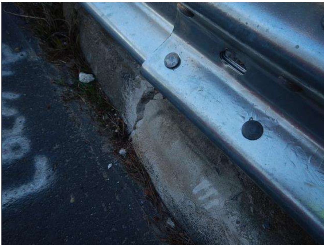
Span 1 Deck: 1 SQUARE FEET SOUND PATCH IN LEFT CURB OVER BENT 1
