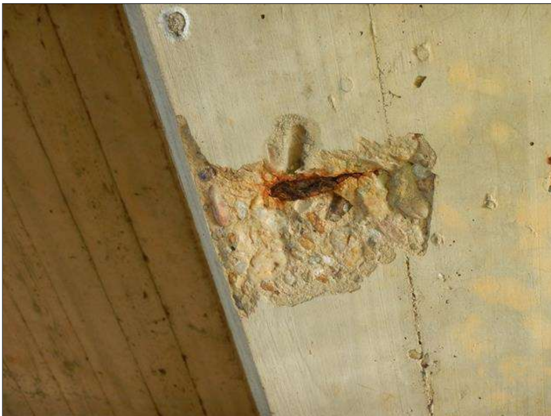
Span 1 Beam 4: 6 INCHES DIAMETER SPALL 3/4 INCHES DEEP WITH EXPOSED STEEL.
