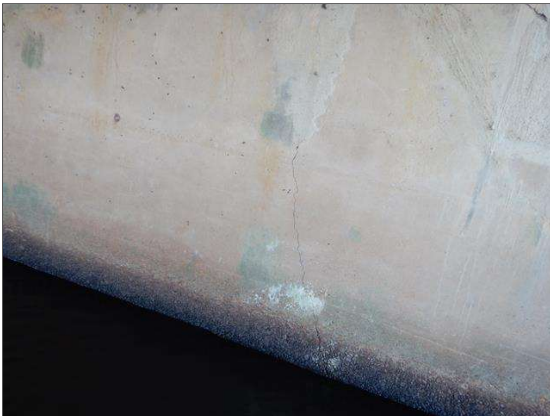
End Bent 1 Abutment: VERTICAL CRACKING 1/16 INCH WIDE IN FACE OF CAP AT GIRDERS 2 & 4 EXTENDING DOWN BREAST WALL.
