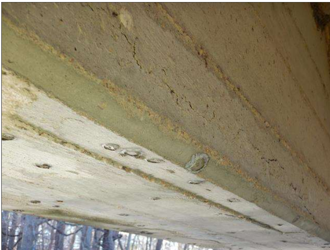
Span 1 Beam 5: 6 INCHES LONG LONGITUDINAL CRACKING IN BOTTOM AND LEFT SIDE AT MID-SPAN.
