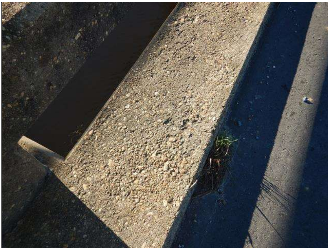
Span 3 Right Bridge Rail: ABRASION ALONG THE RIGHT CURB
