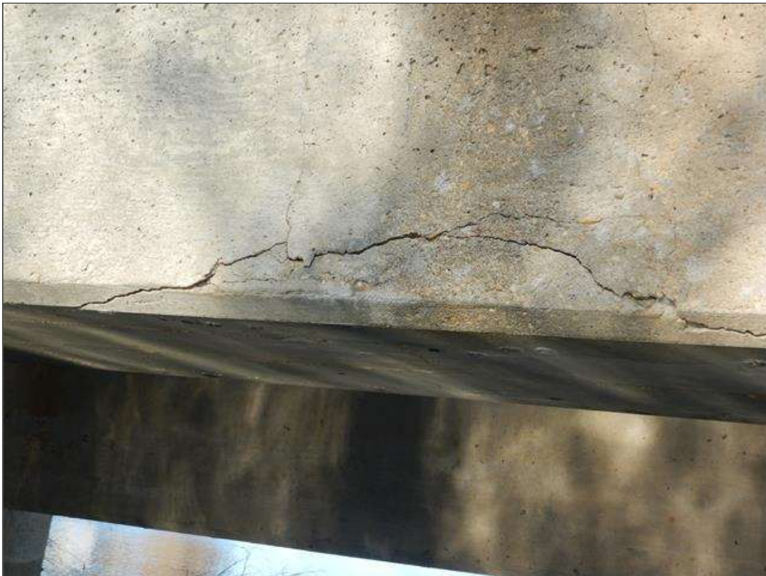
Span 1 Beam 5: 6 FEET CRACKING AND DELAMINATION IN RIGHT SIDE BOTTOM CORNER NEAR MID-SPAN.
