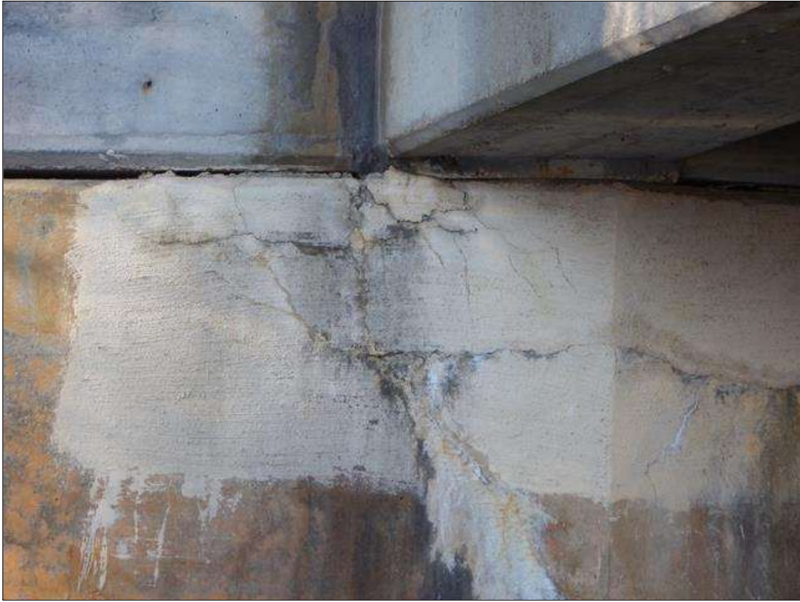
End Bent 1 Abutment: UNSOUND PATCHING IN CAP UNDER GIRDER 5 WITH 1/32 INCH WIDE VERTICAL CRACK IN PATCH.
