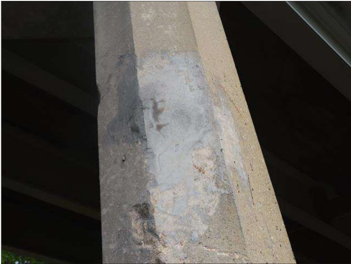
Bent 2 Pile 7: 2 FEET OF PATCHING SPAN 2 SIDE
