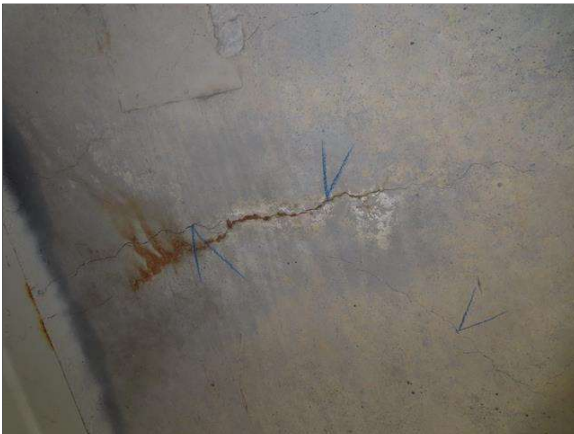
Span 1 Deck: BOTTOM OF DECK: HAIRLINE MAP TRANSVERSE AND DIAGONAL CRACKING IN ALL BAYS
