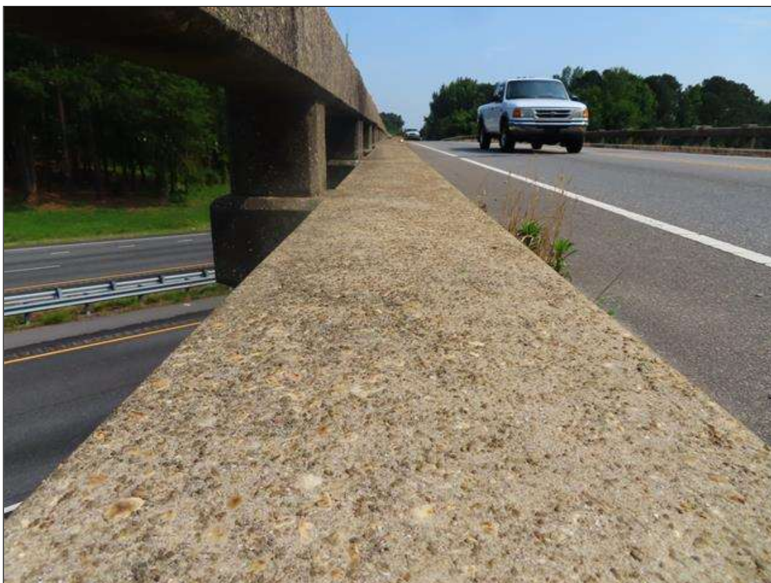
Span 1 Deck: 145 SQUARE FEET OF ABRASION ALONG CURBS.
