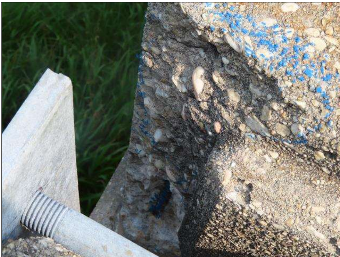
Span 1 Left Bridge Rail: 1 FOOT OF SPALLING IN POST #3. WITH EXPOSED REBAR
