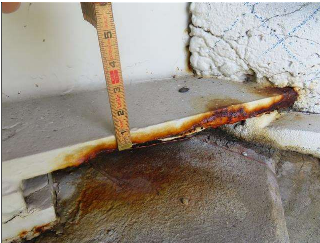
Span 1 Beam 1: SECTION LOSS IN LEFT EDGE BOTTOM FLANGE 4 INCH WIDE 3/4 INCH REMAINING AT END BENT 1
