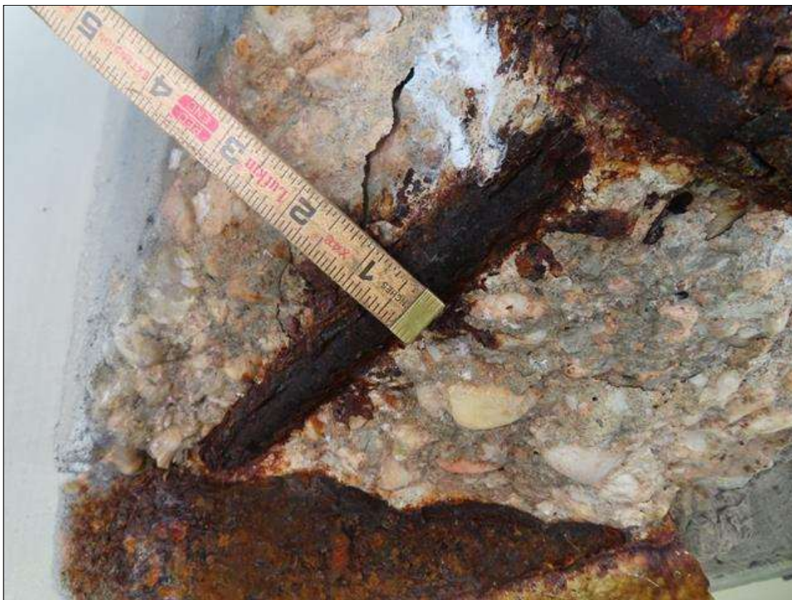
Span 3 Deck: SPALLING AND DELAMINATION WITH SECTION LOSS TO EXPOSED REBAR (ESTIMATED 1 INCH REMAINING) 4 INCHES DEEP X 6 FEET LONG X 10 INCHES WIDE IN SPAN 3 END DIAPHRAGM OVER BENT 3 BAY 2. PAR ISSUED. PHOTO 3 OF 3.
