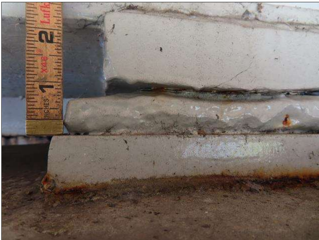
Span 4 Beam 3 Far Bearing: SECTION LOSS ARRESTED, PITTED 1/8 INCH DEEP IN VERTICAL FACES. COATING IS GOOD
