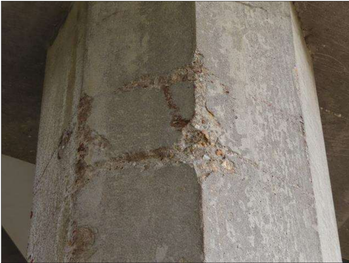
Bent 2 Pile 4: 3 FEET SURFACE SPALLING 1/2 INCH DEEP
