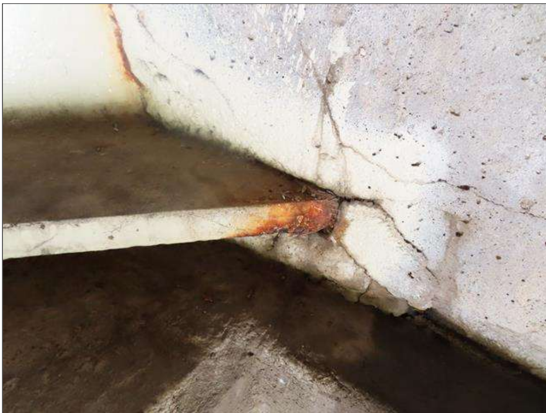
Span 1 Beam 3: FRECKLED RUST
