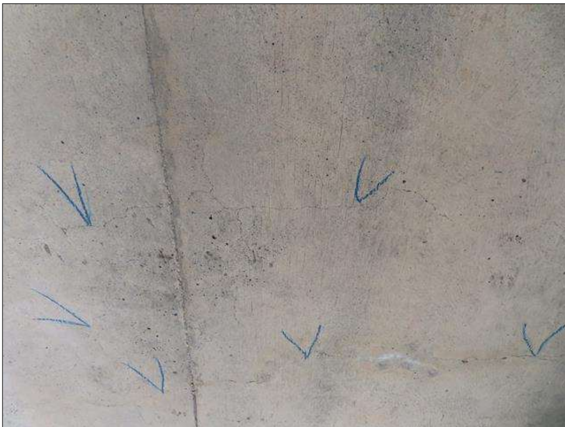
Span 1 Deck: BOTTOM OF DECK: HAIRLINE MAP TRANSVERSE AND DIAGONAL CRACKING IN ALL BAYS
