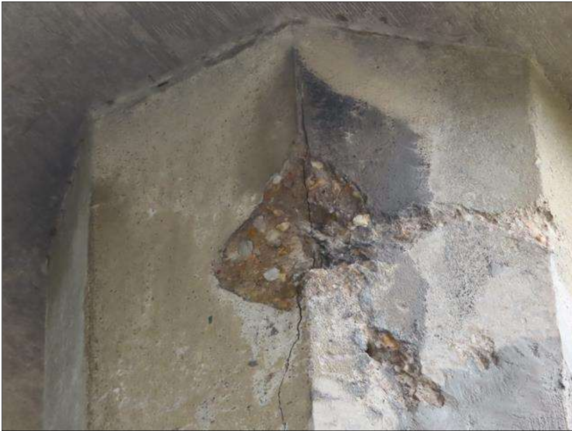
Bent 2 Pile 6: 6 INCH DIAMETER SPALL WITH 1/16 INCH X 1 FEET VERTICAL CRACK SPAN 2 SIDE
