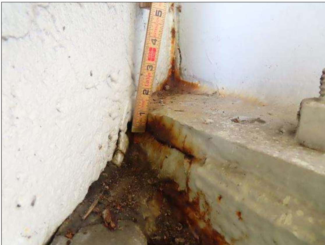
Span 1 Beam 4: SECTION LOSS BOTTOM FLANGE END BENT 1 - 7/8 INCH REMAINING FROM BEARING TO END
