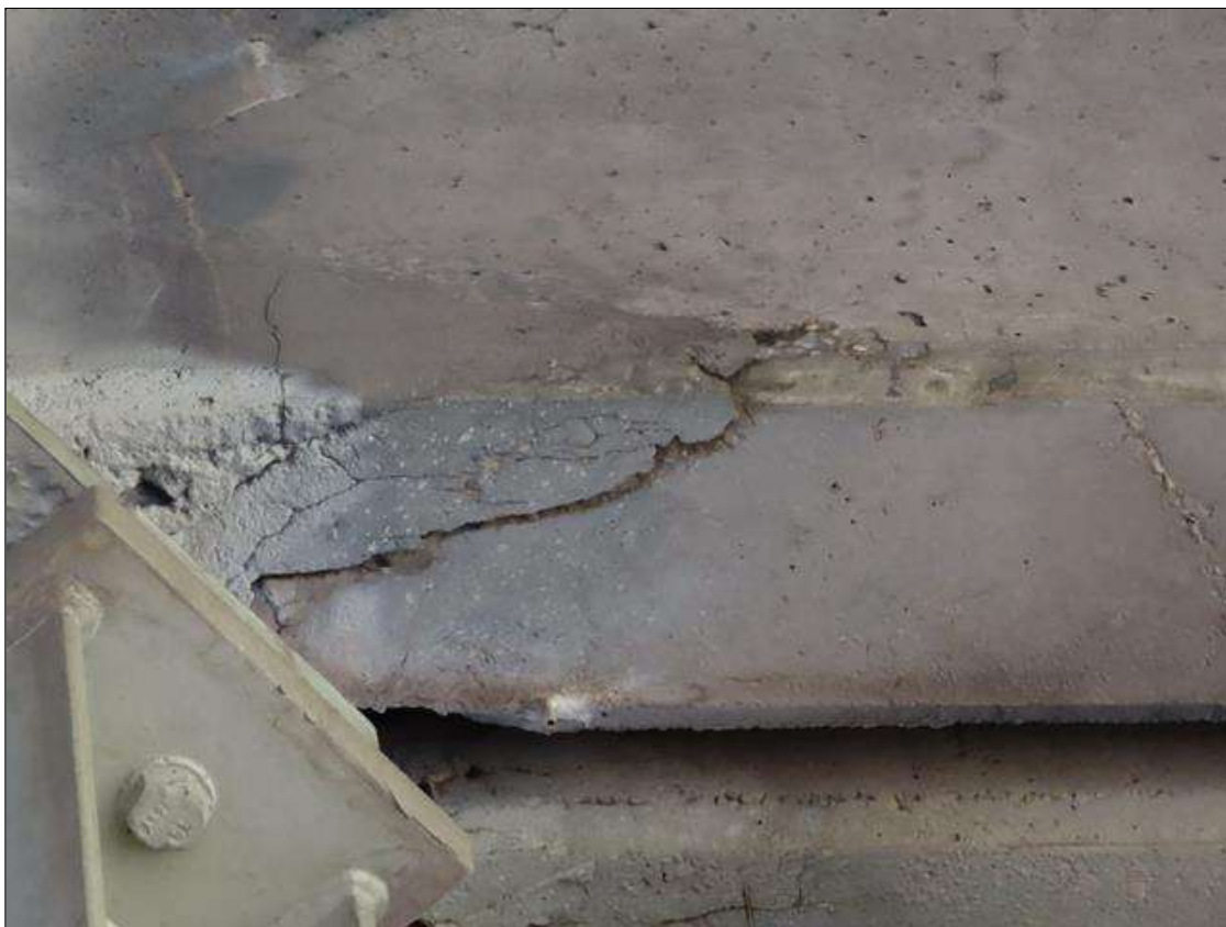
Span 1 Deck: 1/4 INCH WIDE CRACK LEFT OVERHANG DIAPHRAGM, 1 OF FOOT CRACKING IN BAY 1 DIAPHRAGM, 4 FEET OF CRACKING BAY 2 AND 3 DIAPHRAGM
