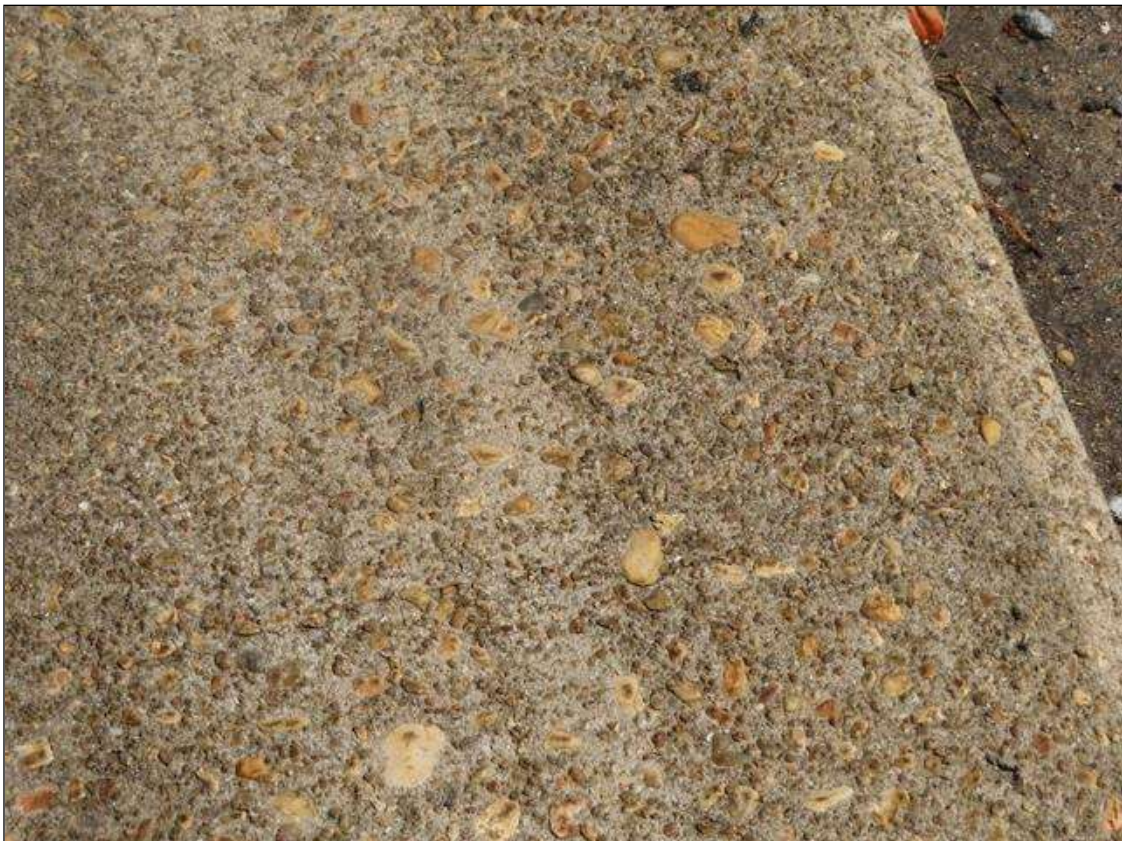
Span 4 Deck: 172 SQUARE FEET OF ABRASION ALONG DECK CURBS.
