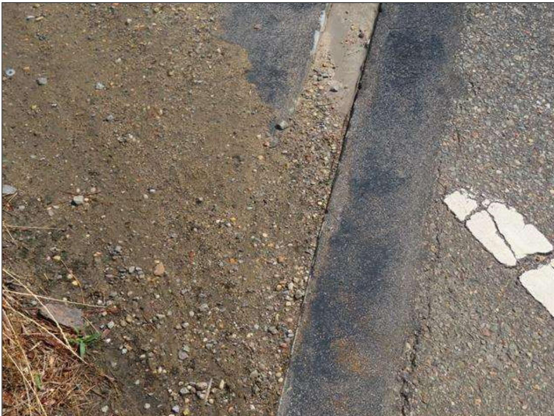
Expansion Joint : DIRT AND DEBRIS IMPACTION
