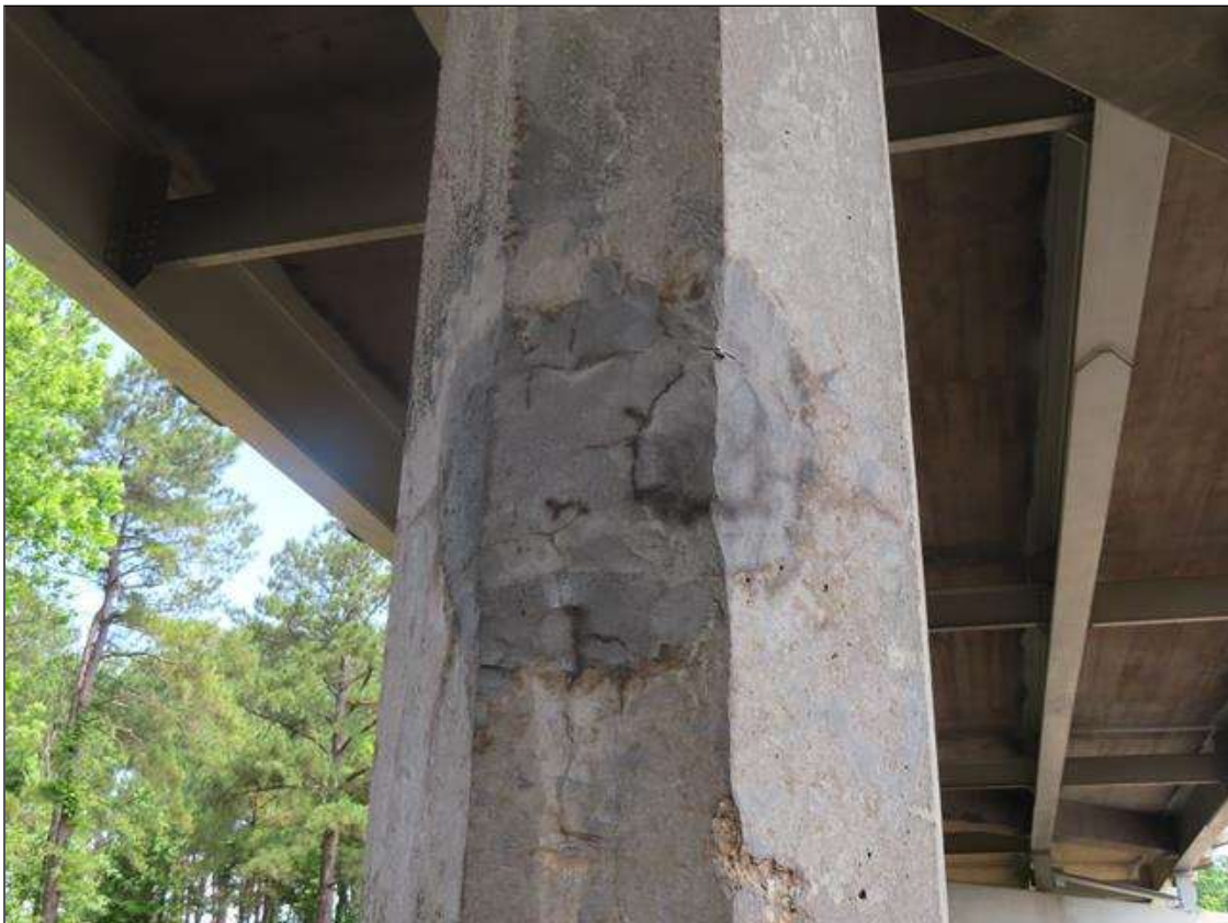
Bent 2 Pile 4: 2 FEET PATCHING
