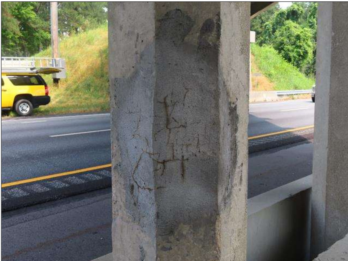
Bent 2 Pile 2: 2 FEET PATCHING
