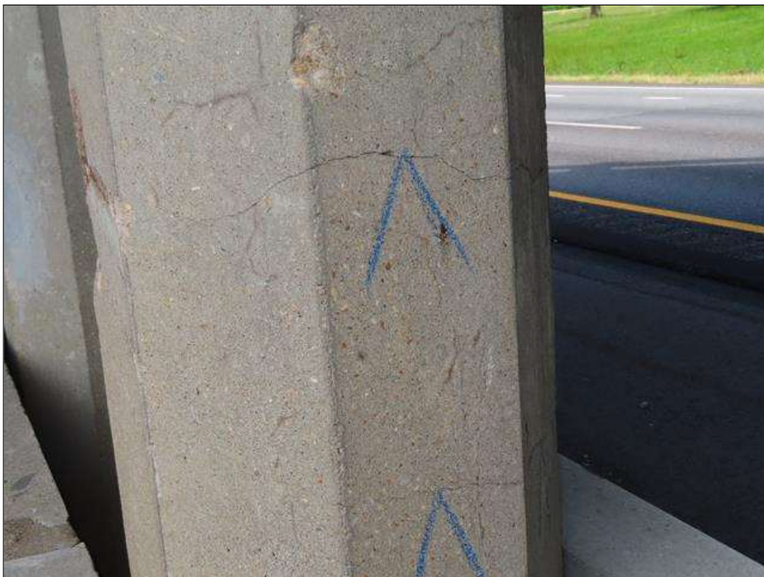
Bent 2 Pile 5: TRANSVERSE CRACKING SPAN 3 SIDE OPPOSITE SPALL IN SPAN 2 SIDE 4 FEET FROM GROUNDLINE
