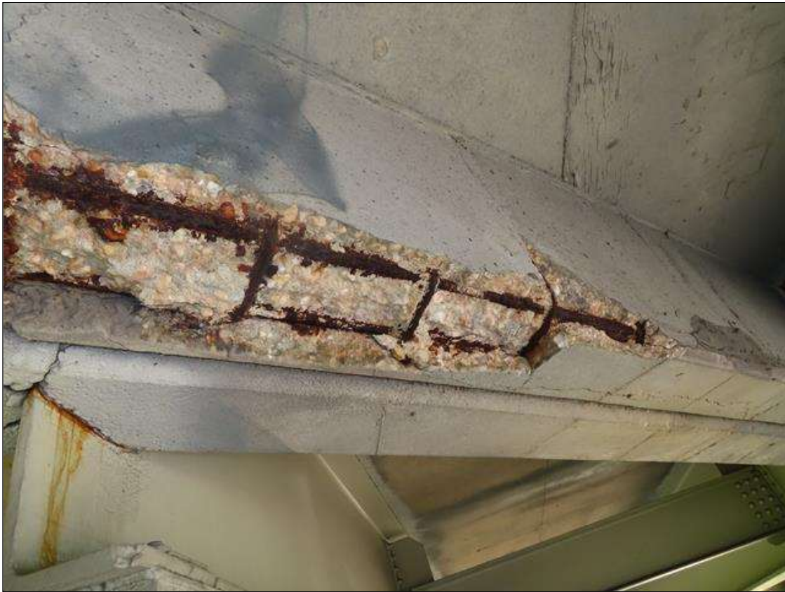
Span 3 Deck: SPALLING AND DELAMINATION WITH SECTION LOSS TO EXPOSED REBAR (ESTIMATED 1 INCH REMAINING) 4 INCHES DEEP X 6 FEET LONG X 10 INCHES WIDE IN SPAN 3 END DIAPHRAGM OVER BENT 3 BAY 2. PAR ISSUED. PHOTO 2 OF 3.
