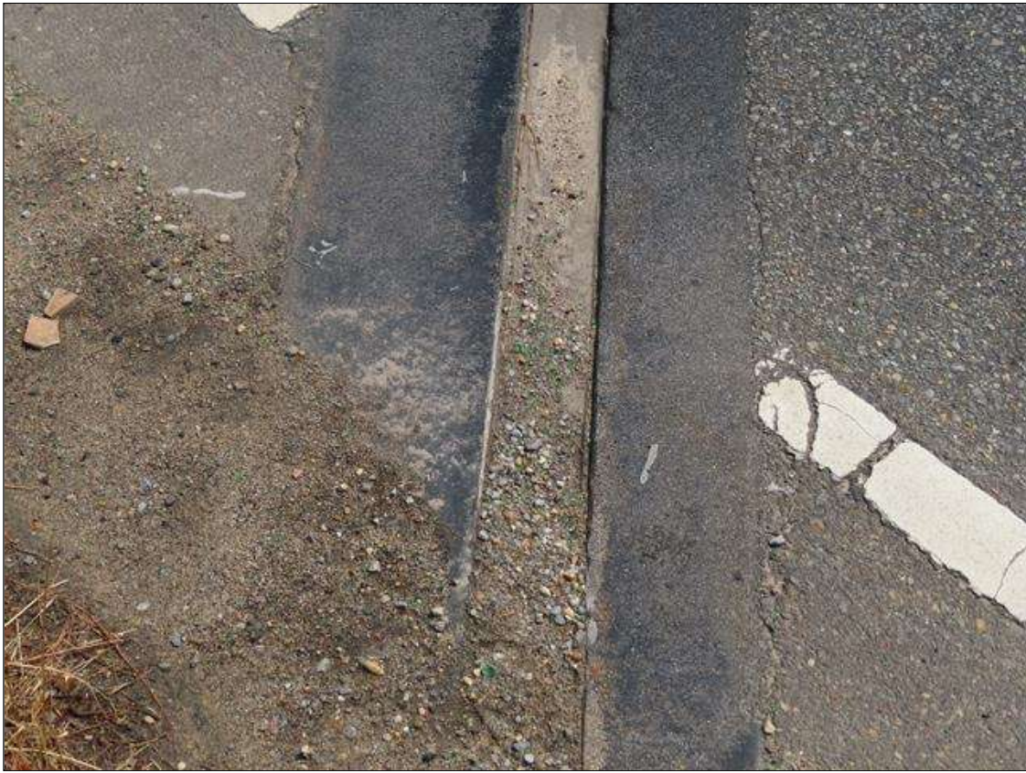
Expansion Joint : DIRT AND DEBRIS IMPACTION
