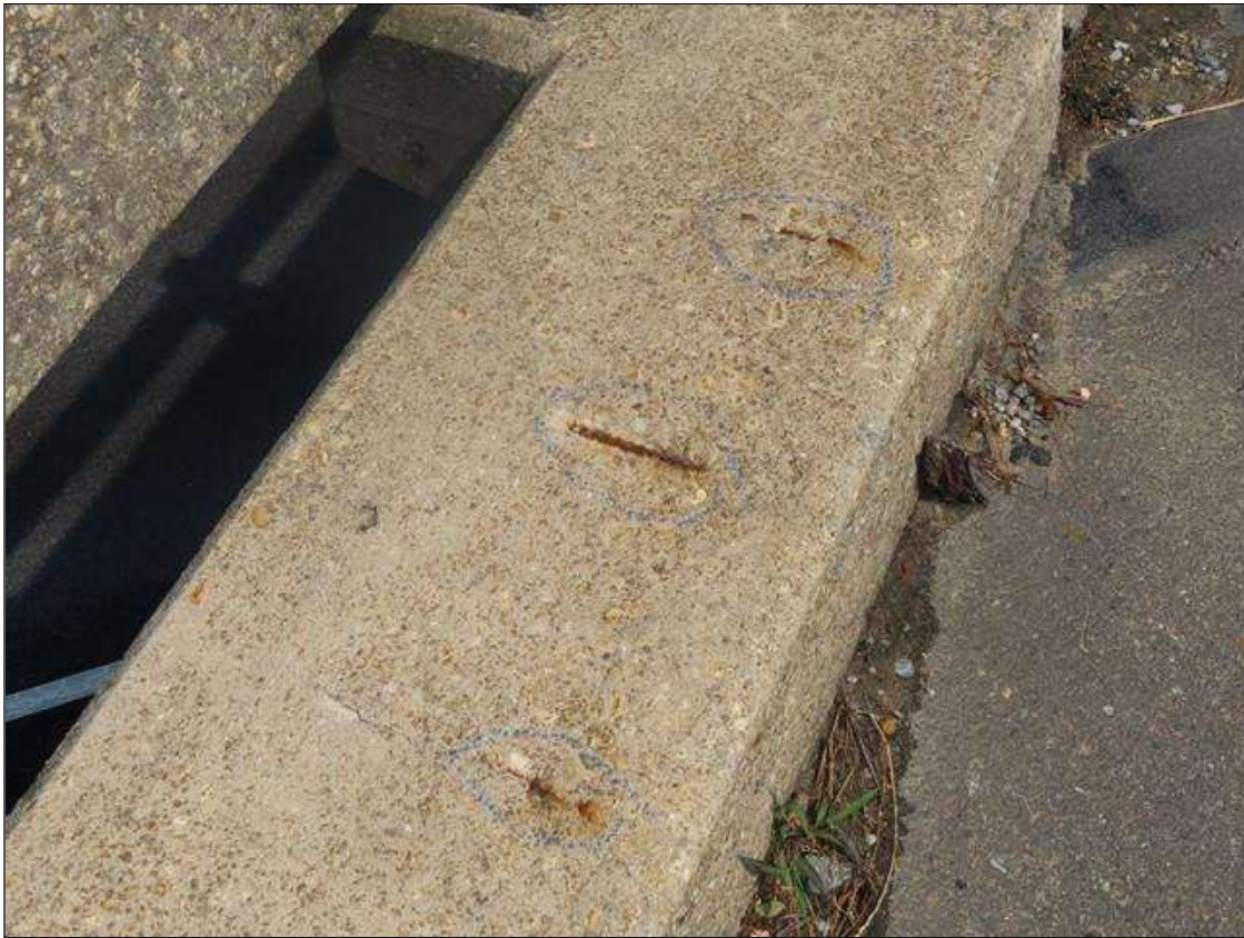
Span 1 Deck: EXPOSED REBAR IN TOP OF CURBING LEFT SIDE
