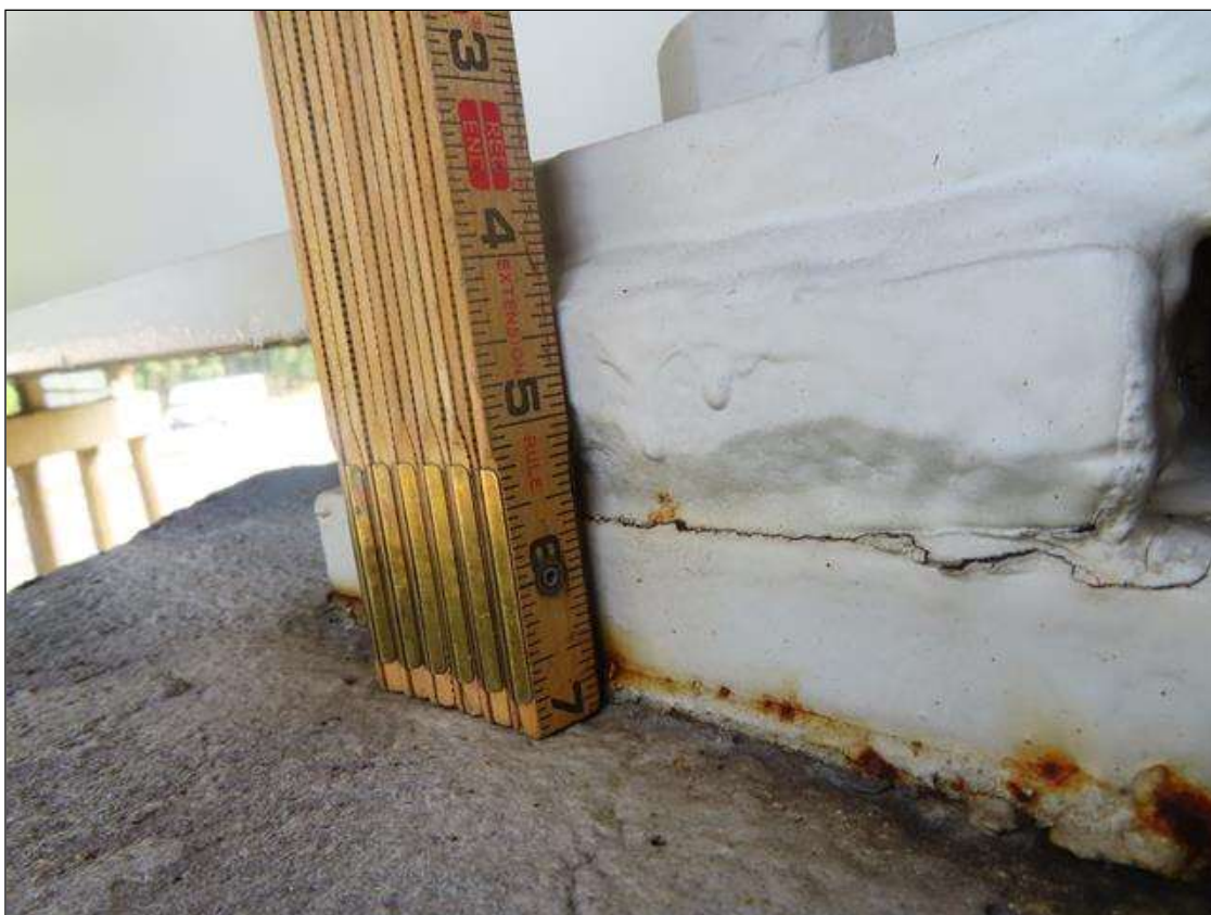
Span 1 Beam 1 Near Bearing: SECTION LOSS ARRESTED , PITTED 1/8 INCH DEEP IN VERTICAL FACES, COATING GOOD
