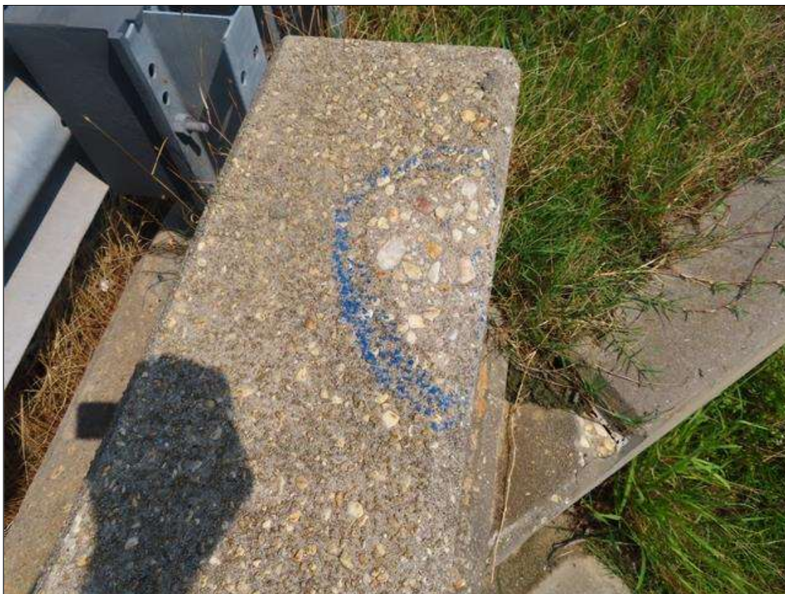
Span 4 Right Bridge Rail: 6 INCH DIAMETER X 1 INCH DEEP SPALL IN END POST
