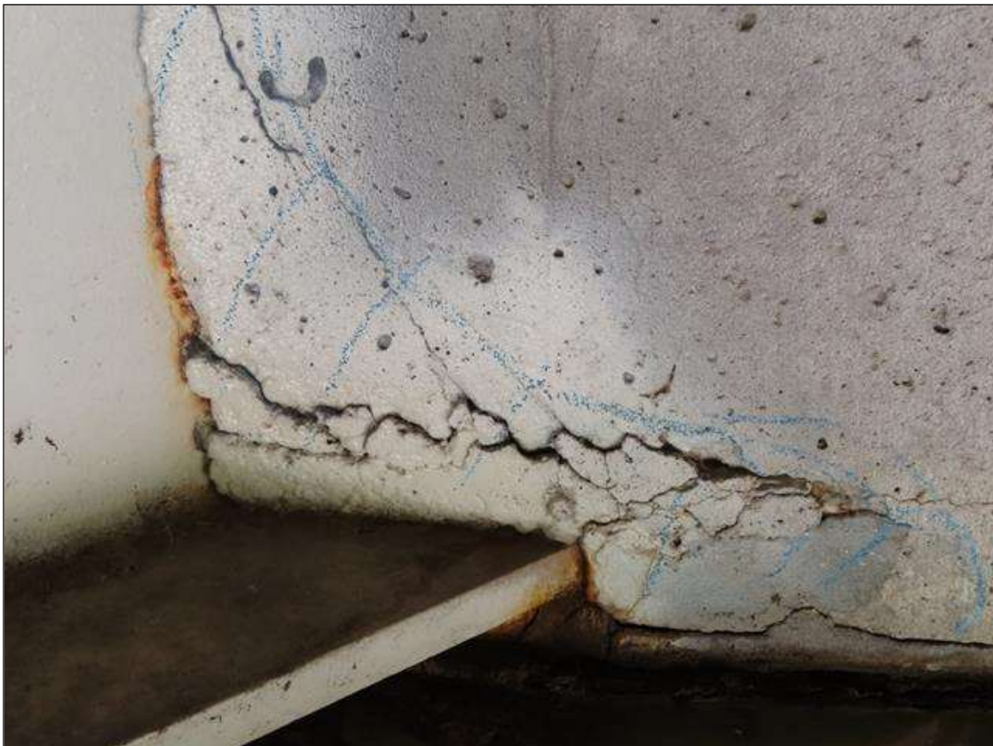
End Bent 1 Cap 1: DELAMINATION IN BE LEFT SIDE BEAM 2 BAY 1
