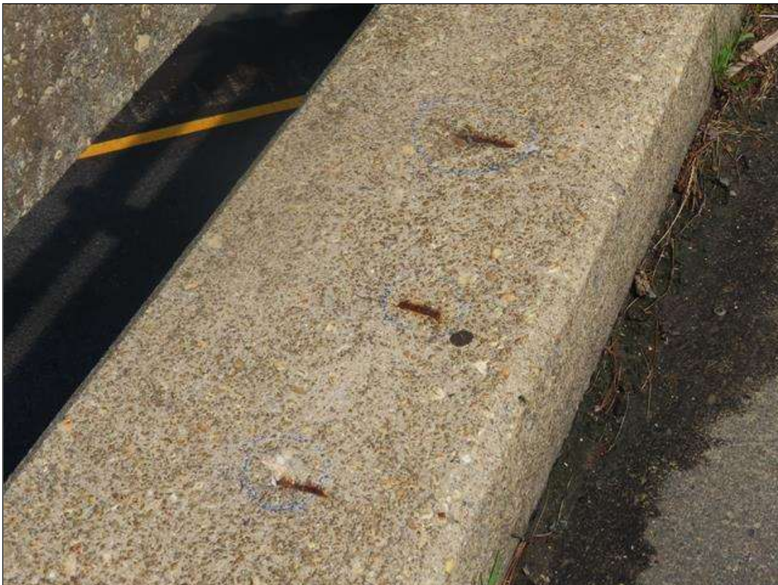
Span 2 Deck: 9 SQUARE FEET OF EXPOSED REBAR ALONG LEFT CURB.
