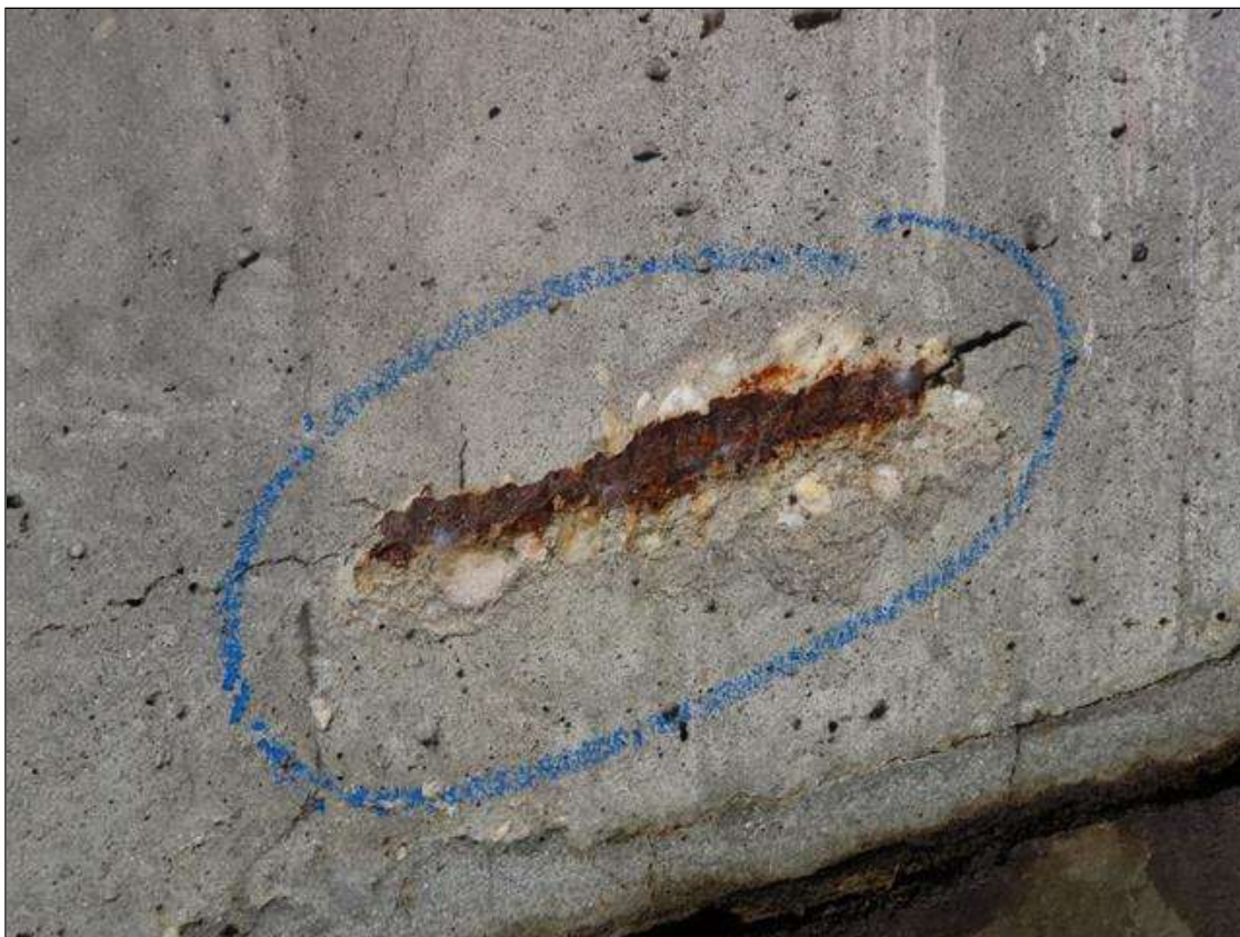
End Bent 2 Abutment/Backwall : 1 FOOT OF EXPOSED REBAR WITH SURFACE SPALLING BAY 2.
