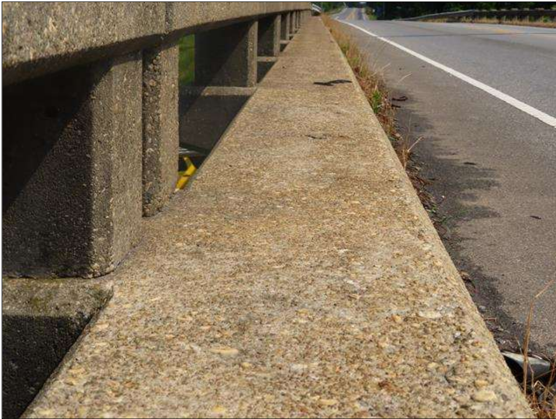
Span 2 Deck: 207 SQUARE FEET OF ABRASION ALONG DECK CURBS.
