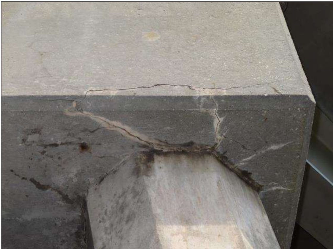
Bent 2 Cap 1: 1/32 INCH CRACKS RADIATING BOTTOM OF CAP AT PILE 7
