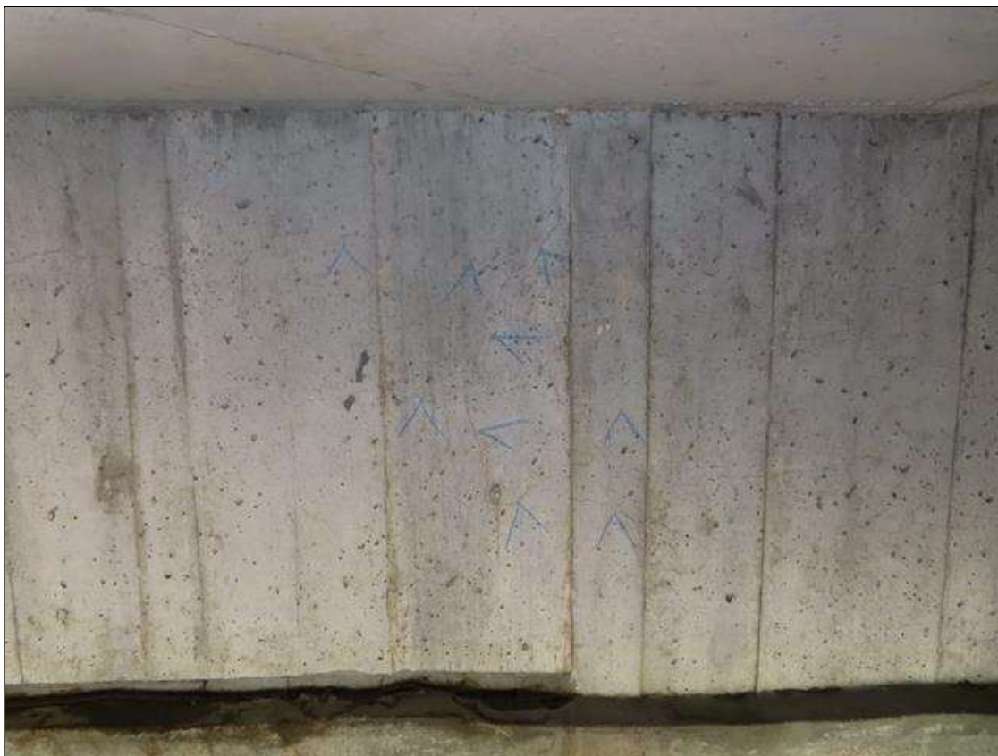
End Bent 1 Abutment/Backwall : ALL BAYS HAVE HAIRLINE MAP CRACKING
