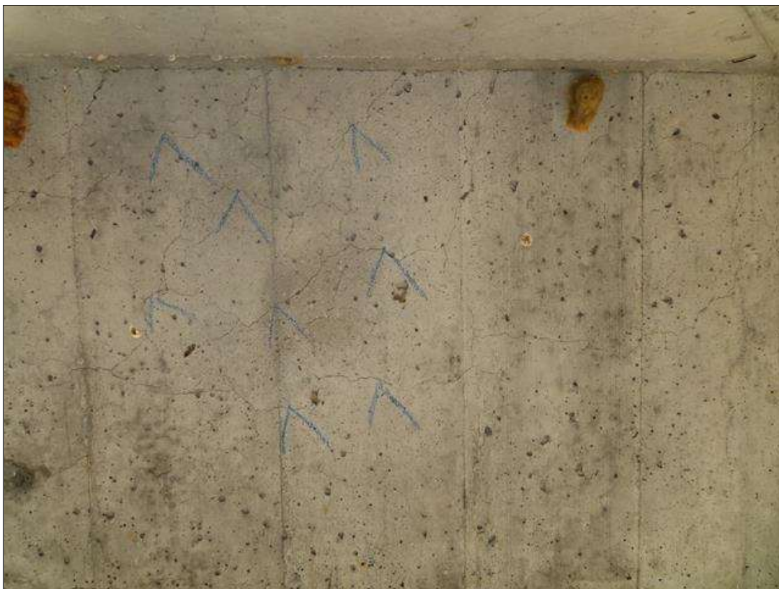
End Bent 2 Abutment/Backwall : 28 FEET HAIRLINE MAP CRACKING FULL LENGTH
