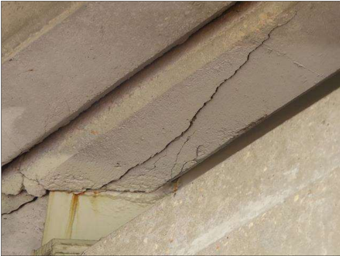
Span 3 Deck: 4 FEET TRANSVERSE CRACKING IN OVERHANGS AND TRANSVERSE CRACKING BENT 2 DIAPHRAGMS
