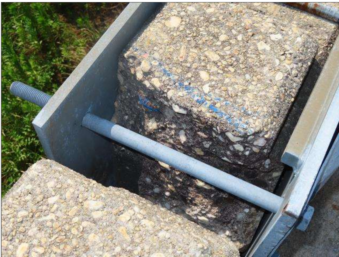
Span 1 Right Bridge Rail: 1 FOOT OF SPALL WITH EXPOSED REBAR IN POST #2.
