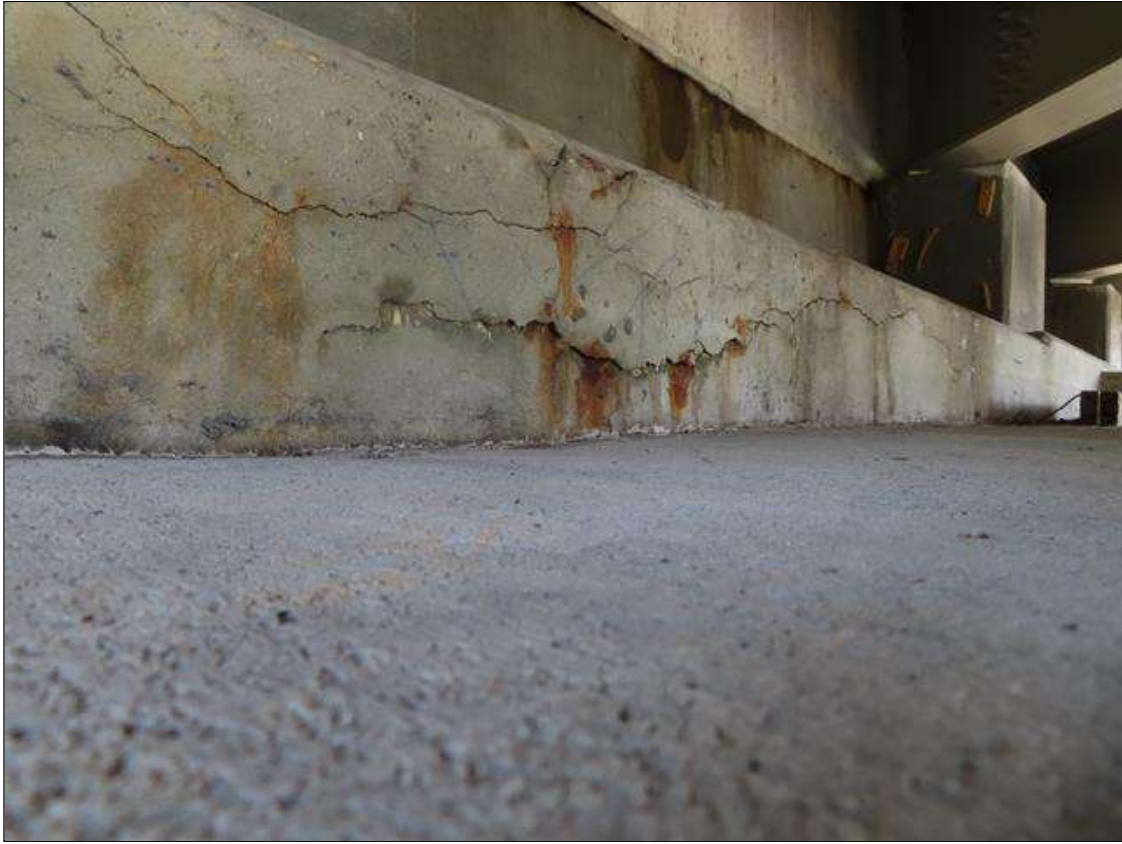
End Bent 2 Cap 1: 8 FEET LONGITUDINAL CRACKING FACE AND TOP OF CAP WITH DELAMINATION BETWEEN AND RUST STAINING UNDER BAY 1
