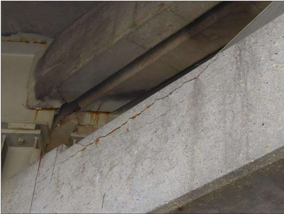
Bent 1 Cap 1: 8 FEET OF 1/4 INCH LONGITUDINAL CRACKING WITH RUST STAINING SPAN 2 SIDE UNDER BAY
