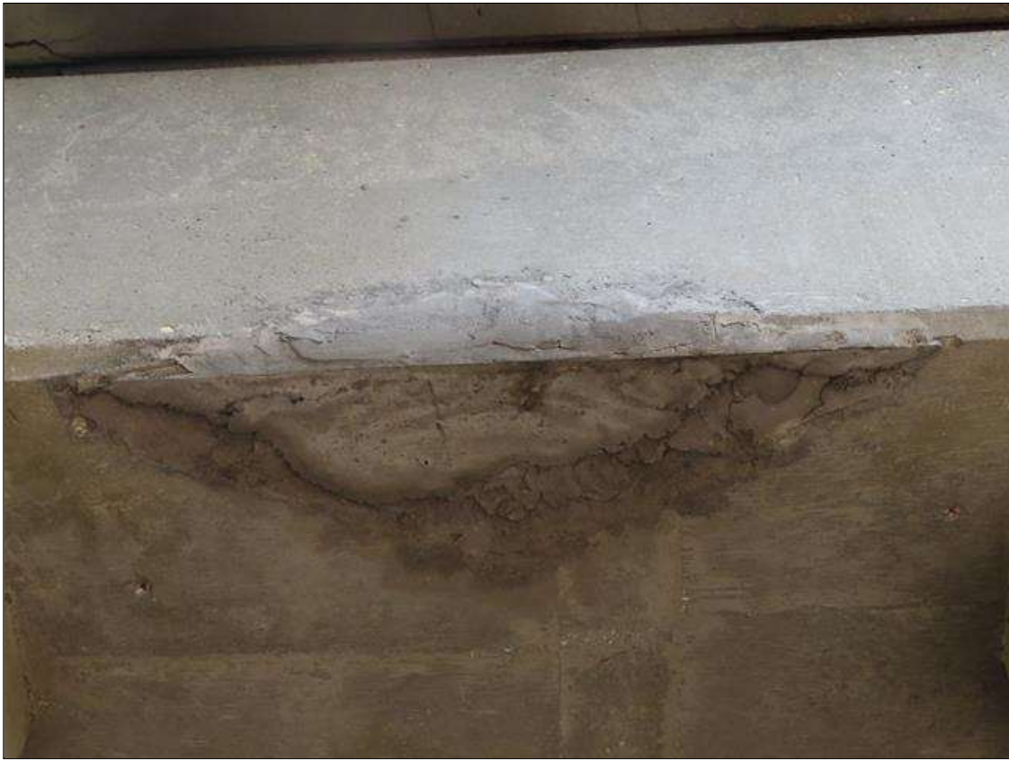
Bent 2 Cap 1: 3 FEET OF PATCHING BOTTOM OF CAP UNSOUND BAY 3
