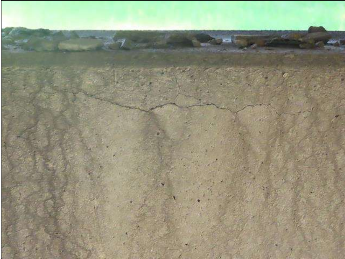
Bent 1 Cap 1: 3 FEET OF 1/16 INCH LONGITUDINAL CRACK BAY 1 SPAN 1 SIDE
