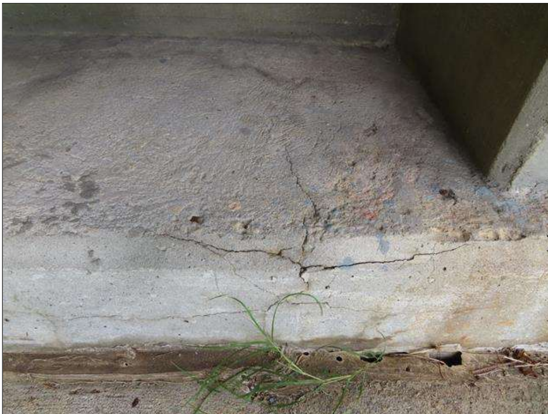
End Bent 1 Cap 1: 3 FEET CRACKING BAY 1 TOP , FACE 1/16 INCH WIDE
