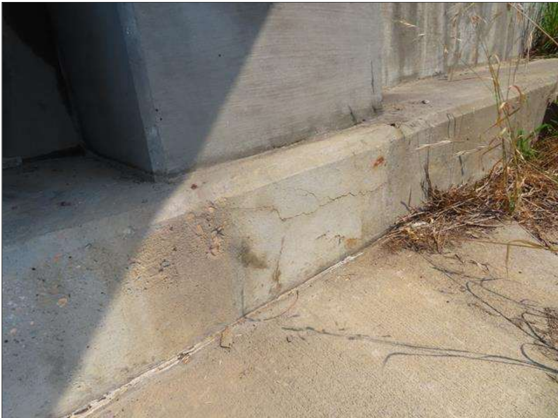
End Bent 2 Cap 1: 3 FEET X 1/8 INCH LONGITUDINAL FACE OF CAP BEAM 4
