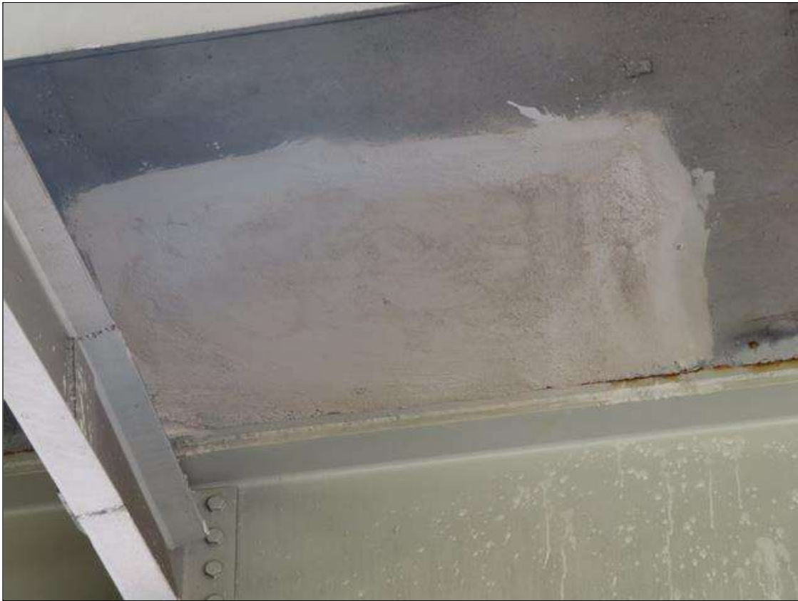
Span 2 Deck: 10 SQUARE FEET OF SOUND PATCHING IN BOTTOM OF DECK BAY 1 AT 1/3 POINT FROM BENT 1. THIS AREA WAS PREVIOUSLY DELAMINATING OVER LANES OF TRAFFIC AND WAS ISSUED A PRIORITY MAINTENANCE AND HAS BEEN REPAIRED SINCE LAST INSPECTION.
