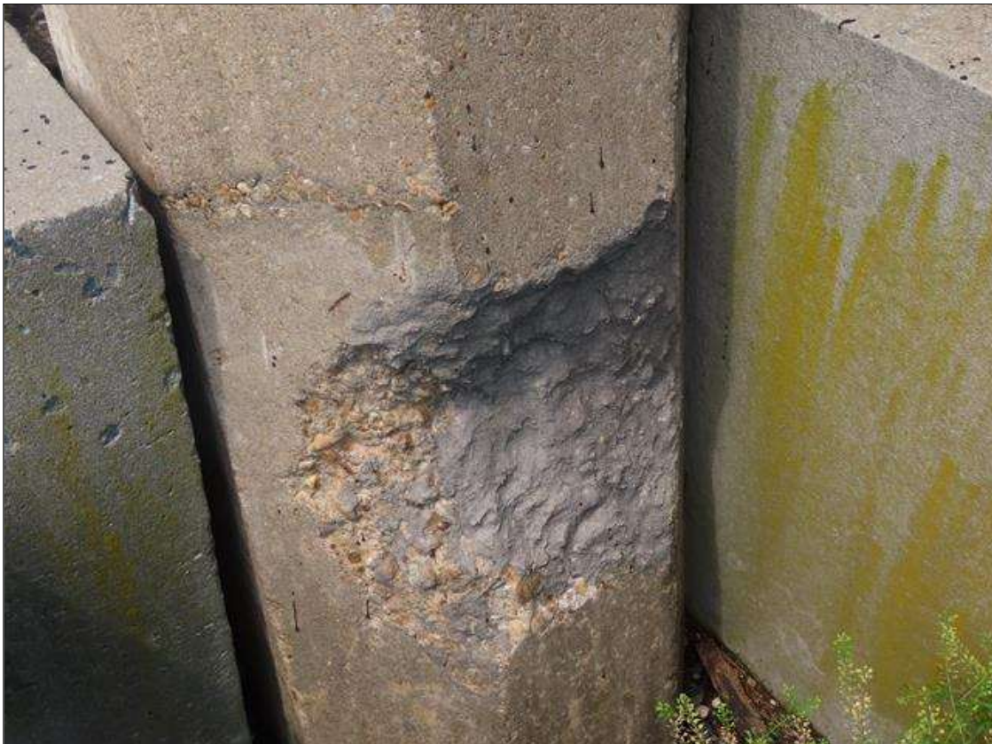
Bent 2 Pile 7: SPALL 1 FOOT FROM GROUNDLINE 4 INCH DEEP X 16 INCH DIAMETER RIGHT SIDE WITH 3 1/32 INCH HORIZONTAL CRACKS LEFT SIDE OPPOSITE SPALL
