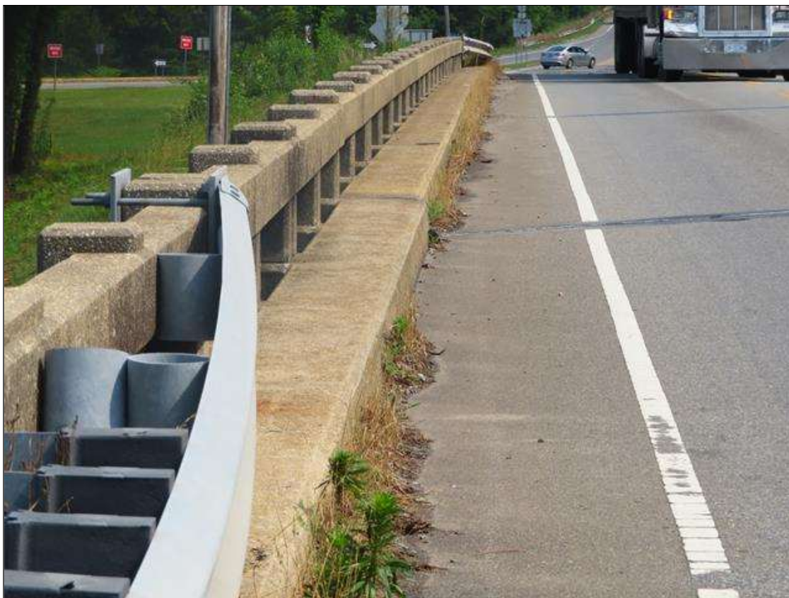
VEGETATION WITH DIRT AND DEBRIS OUT 1.5 FEET IN SHOULDERS.
