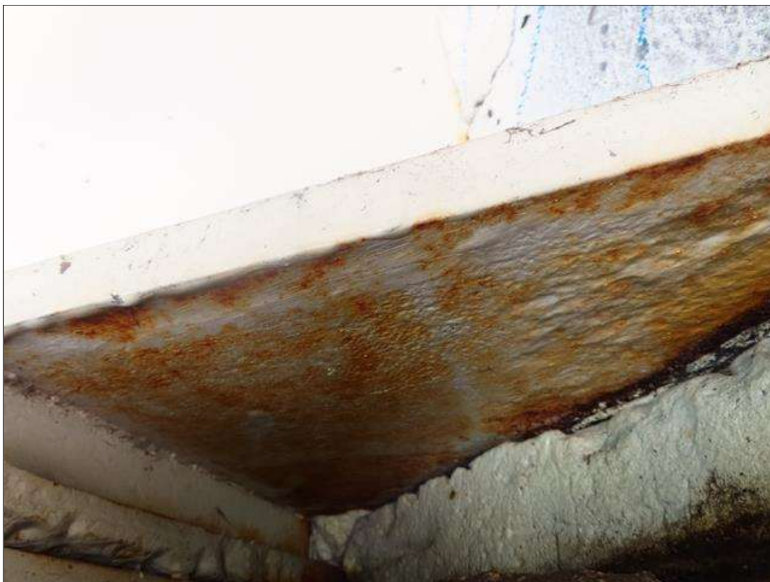
Span 4 Beam 3: SURFACE RUST BOTTOM FLANGE
