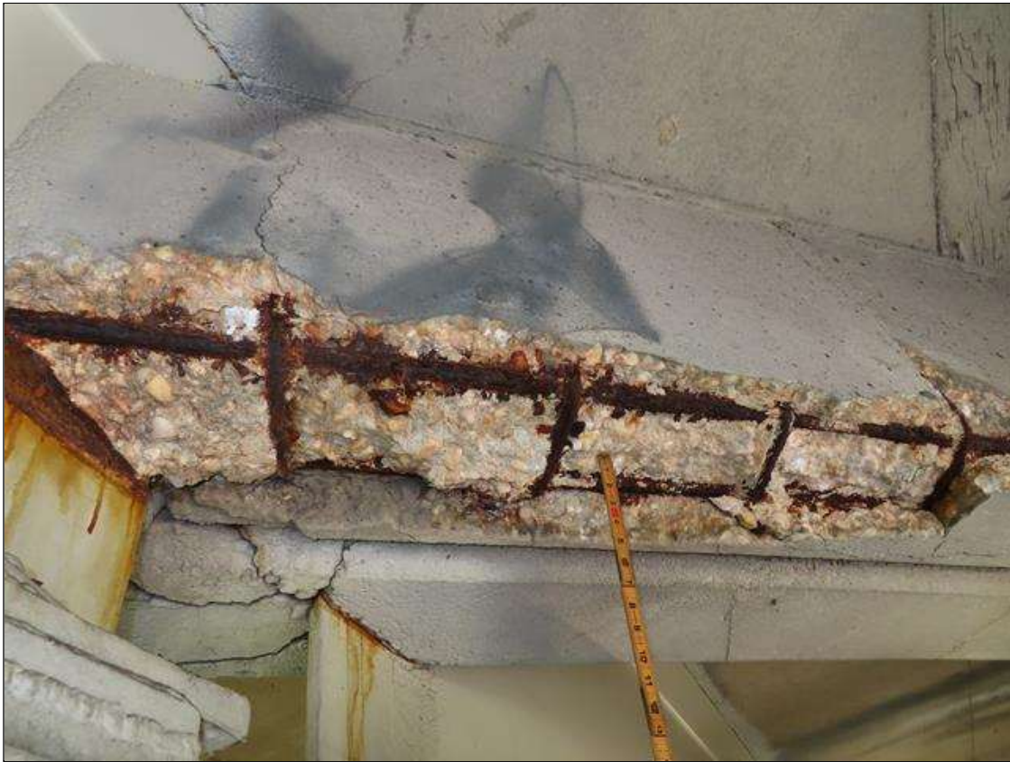
Span 3 Deck: SPALLING AND DELAMINATION WITH SECTION LOSS TO EXPOSED REBAR (ESTIMATED 1 INCH REMAINING) 4 INCHES DEEP X 6 FEET LONG X 10 INCHES WIDE IN SPAN 3 END DIAPHRAGM OVER BENT 3 BAY 2. PAR ISSUED. PHOTO 1 OF 3.
