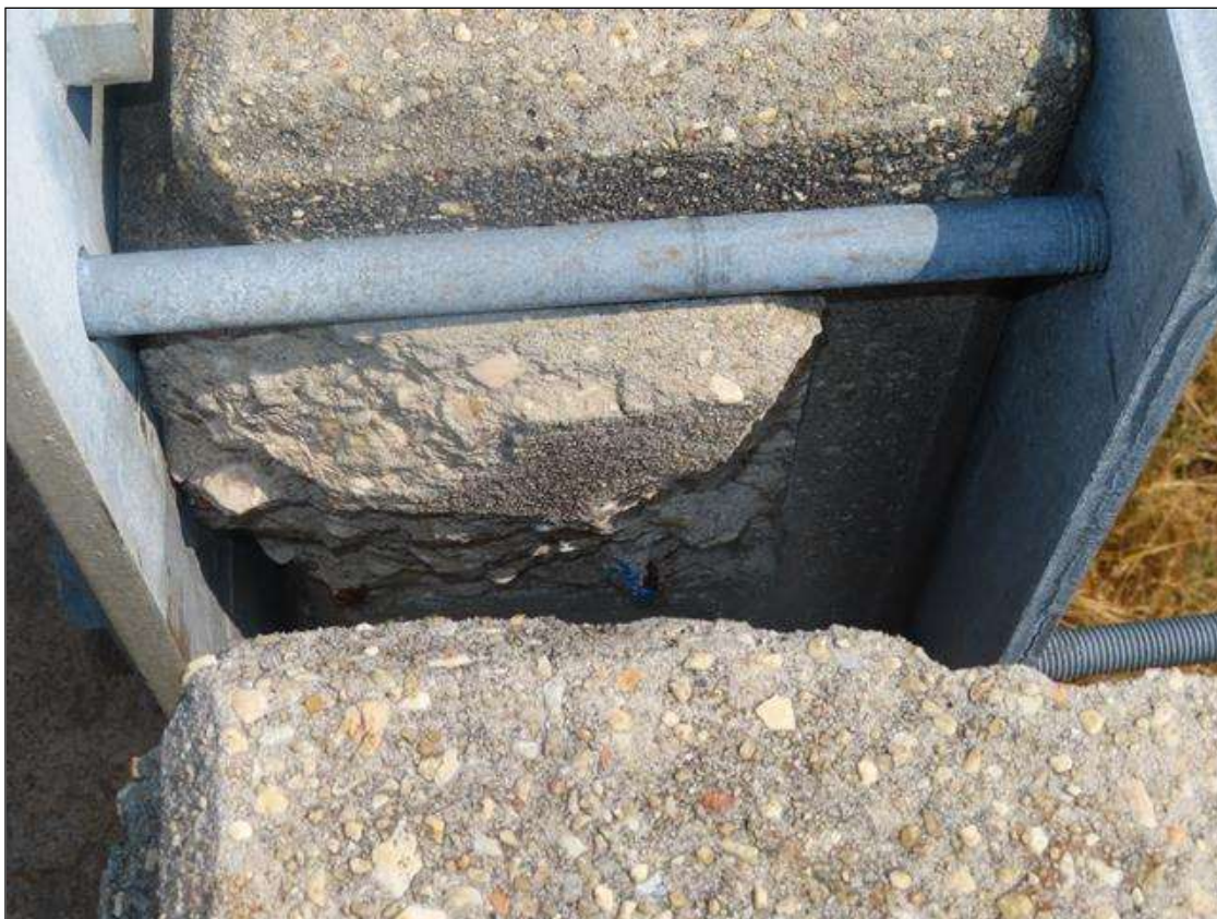
Span 4 Right Bridge Rail: 1 FOOT OF SPALLING WITH EXPOSED REBAR IN POST #6.
