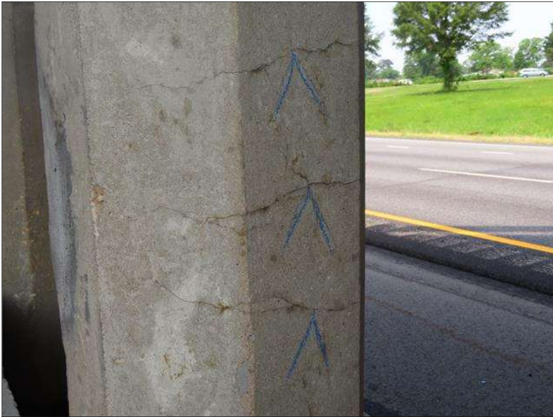
Bent 2 Pile 2: 3 TRANSVERSE 1/32 INCH CRACKS RIGHT SIDE 4 FEET FROM GROUNDLINE
