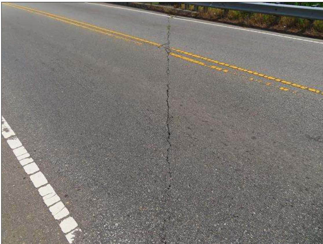
Span 1 Wearing Surface: 28 SQUARE FEET OF CRACKING OVER END BENT 1.
