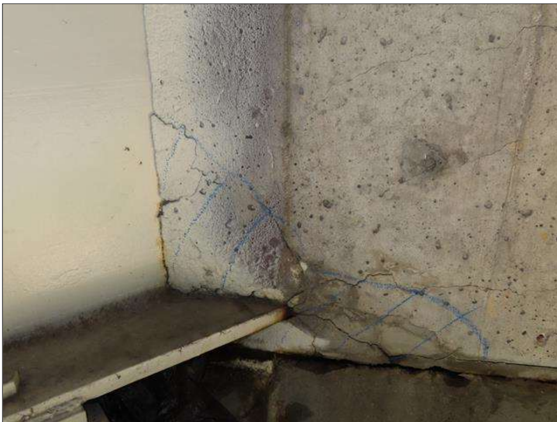
End Bent 2 Abutment/Backwall : 4 FEET DELAMINATION IN ALL BAYS ADJACENT TO BEAMS.
