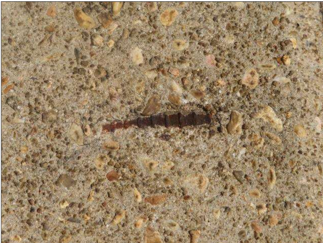
Span 3 Deck: 1 SQUARE FEET OF EXPOSED REBAR IN THE LEFT CURB.
