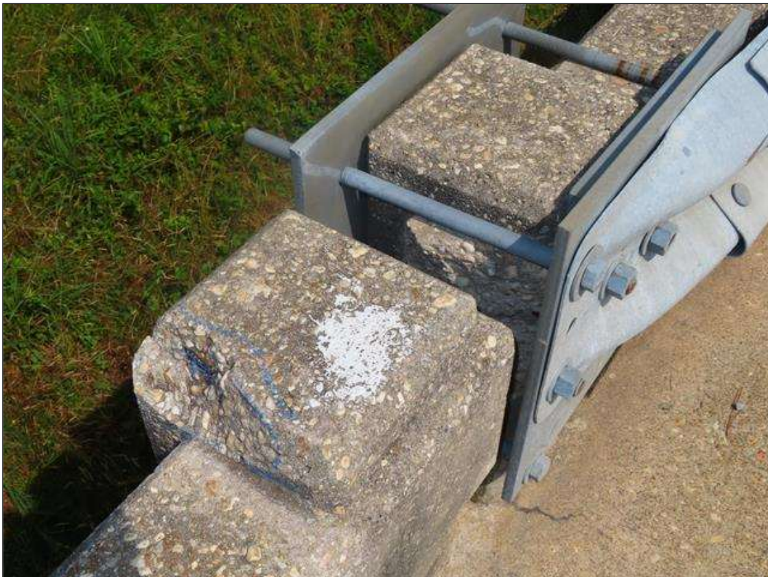
Span 4 Left Bridge Rail: 2 FEET OF SPALLING IN POSTS 5 & 6. WITH EXPOSED REBAR
