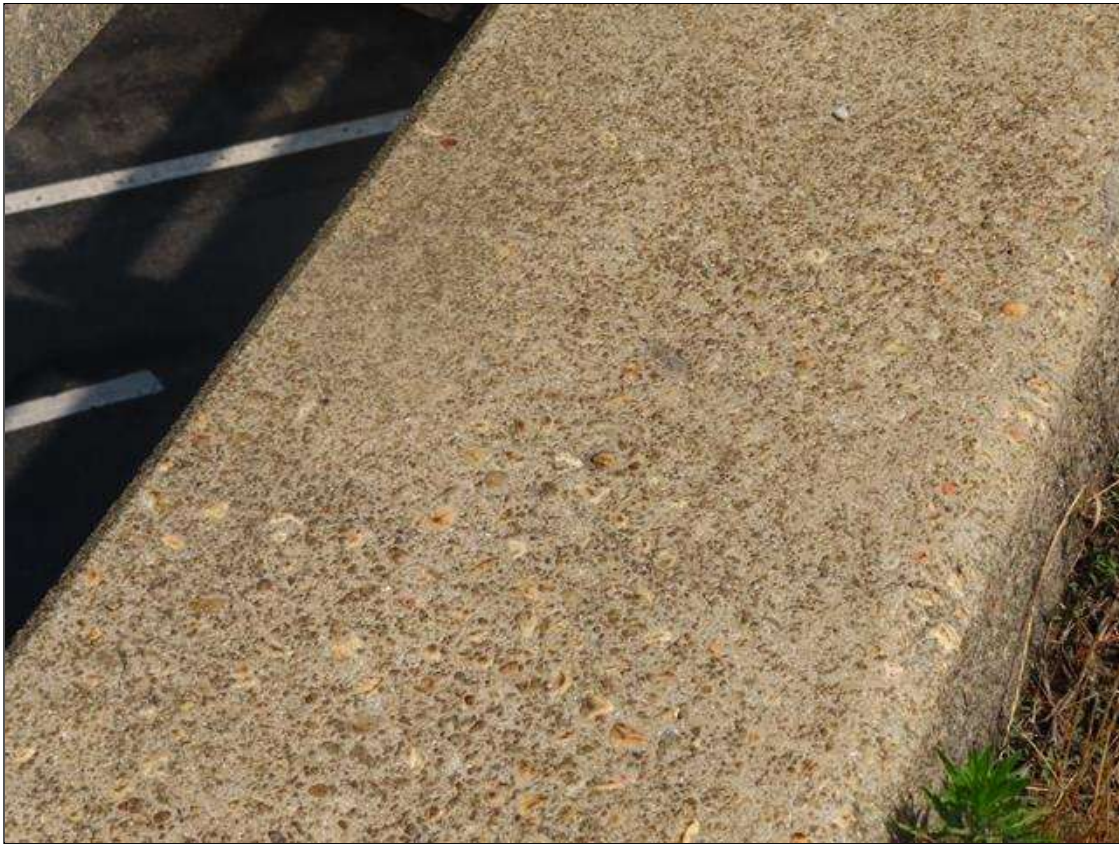
Span 3 Deck: 216 SQUARE FEET OF ABRASION ALONG DECK CURBS.
