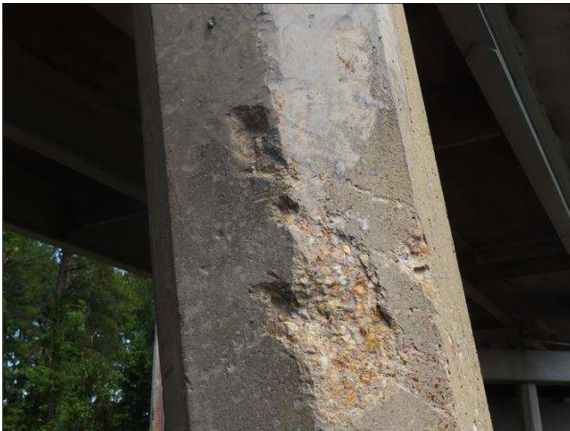
Bent 2 Pile 7: 2 FEET SPALLING SPAN 2 SIDE
