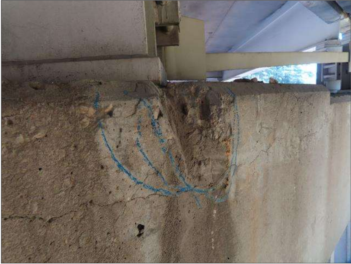
Bent 3 Cap 1: 6 INCH DIAMETER SPALL SPAN 4 SIDE 1 INCH DEEP TOP CORNER BEAM 2
