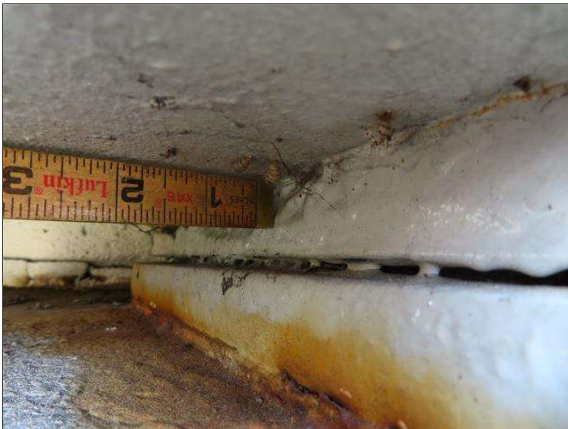
Span 4 Beam 4 Far Bearing: SECTION LOSS ARRESTED, PITTED 1/8 INCH DEEP IN VERTICAL FACES AND FRECKLED RUST
