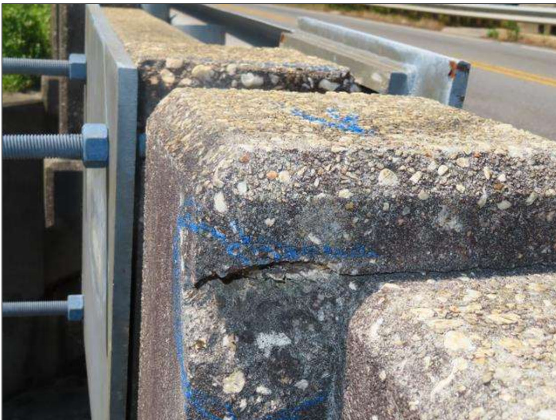
Span 1 Right Bridge Rail: 1 FOOT OF SPALLING WITH CRACKING IN POST #3.
