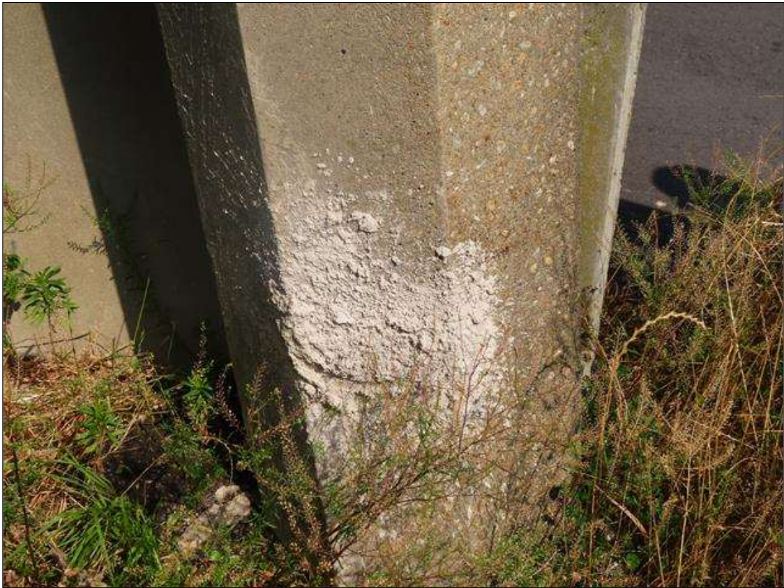
Bent 1 Pile 6: 5 FEET OF PATCHING
