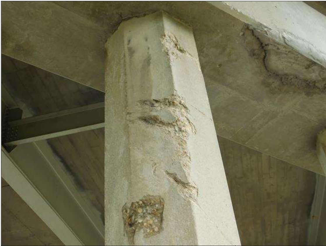
Bent 2 Pile 5: 5 SPALLS 1 IN DEEP TOTALLING 6 SQUARE FEET
