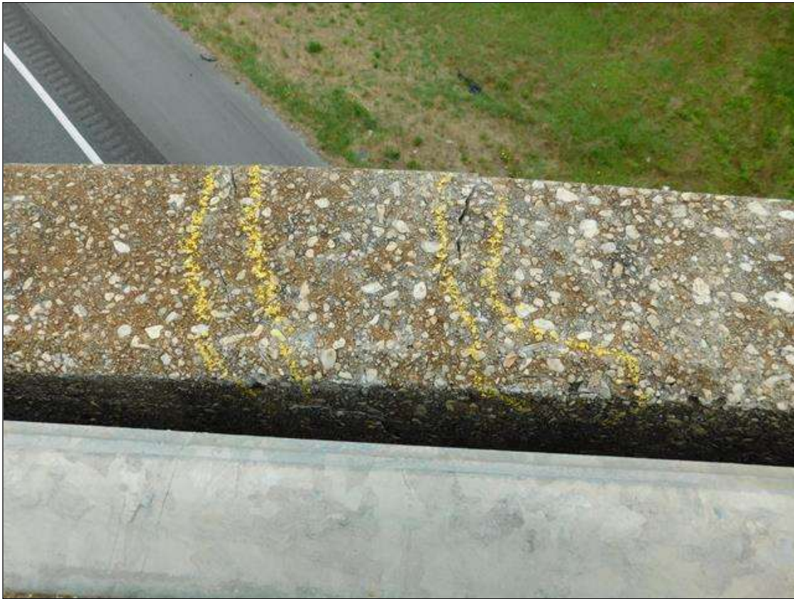
Span 2 Right Bridge Rail: IMPACT DAMAGE. THE 4TH GUARDRAIL POST FROM BENT 1 IS CRACKED, SPALLED AND LEANING OUT 1.5" AT TOP (REFERENCED FROM POST 3). HORIZONTAL RAILING FROM POST 4 TO POST 5 IS CRACKED AND PUSHED OUT. POSTS 5 & 6 HAVE WRAP-AROUND CRACKING AT BOTTOM OF POSTS BUT APPEAR TO BE PLUMB. TEMPORARY STEEL GUARDRAIL HAS BEEN ADDED FROM POST 3 TO POST 7. AFFECTED AREA IS OVER THE NORTHBOUND LANES OF I-95. PAR ISSUED.
