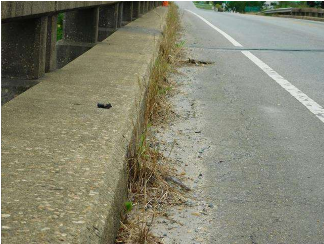
DIRT AND VEGETATION ALONG CURBLINES
