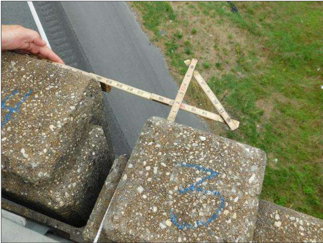
Span 2 Right Bridge Rail: IMPACT DAMAGE. THE 4TH GUARDRAIL POST FROM BENT 1 IS CRACKED, SPALLED AND LEANING OUT 1.5" AT TOP (REFERENCED FROM POST 3). HORIZONTAL RAILING FROM POST 4 TO POST 5 IS CRACKED AND PUSHED OUT. POSTS 5 & 6 HAVE WRAP-AROUND CRACKING AT BOTTOM OF POSTS BUT APPEAR TO BE PLUMB. TEMPORARY STEEL GUARDRAIL HAS BEEN ADDED FROM POST 3 TO POST 7. AFFECTED AREA IS OVER THE NORTHBOUND LANES OF I-95. PAR ISSUED.
