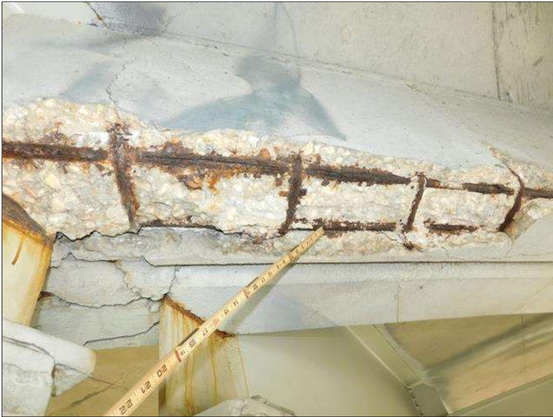
Span 3 Deck: 6' OF SPALLING AND DELAMINATION WITH SECTION LOSS TO EXPOSED REBAR (ESTIMATED 1 INCH REMAINING) 4 INCHES DEEP X 6 FEET LONG X 10 INCHES WIDE IN SPAN 3 END DIAPHRAGM OVER BENT 3, BAY 2. PAR ISSUED.
