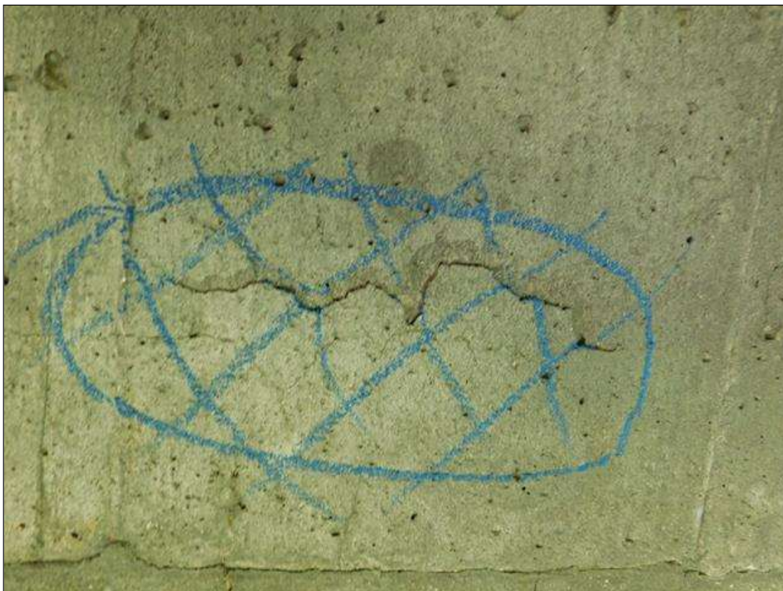
End Bent 2 Abutment: DELAMINATION IN BAY 2 ADJACENT TO EXPOSED REBAR.
