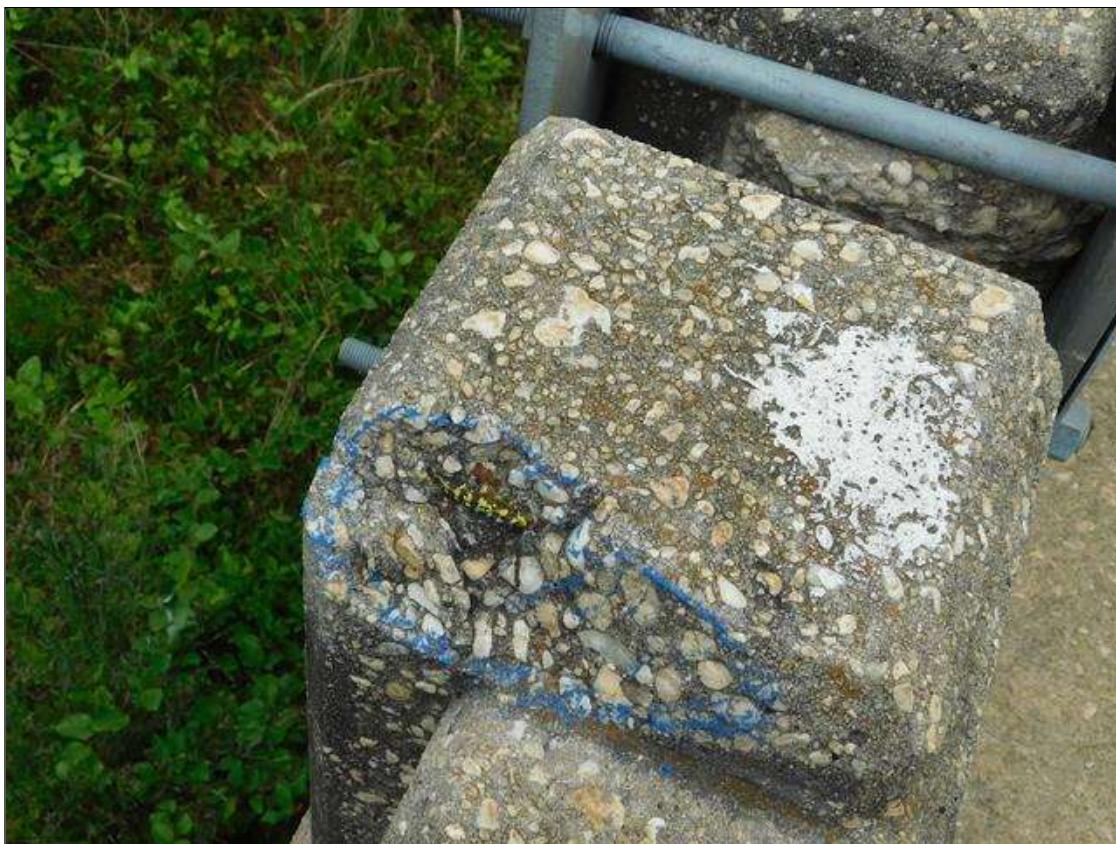
Span 4 Left Bridge Rail: 2 FEET OF SPALLING IN POSTS 5 & 6. WITH EXPOSED REBAR.
