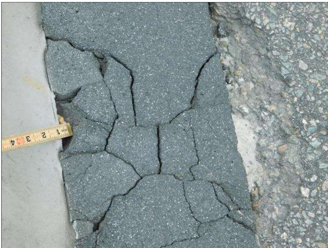
Span 2 Wearing Surface: CRACKING IN ELASTOMERIC CONCRETE OVER THE SOUTHBOUND LANE.
