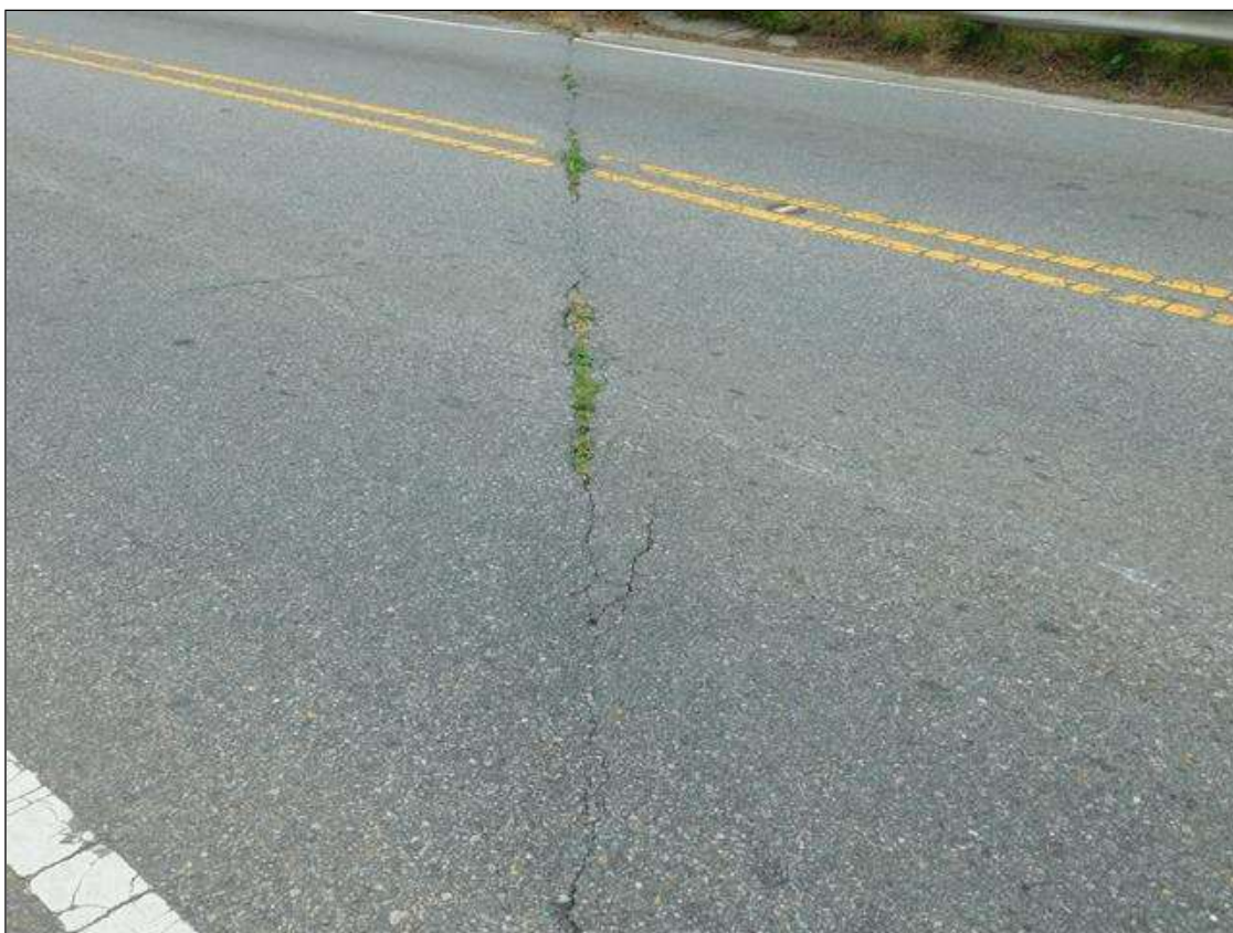
Span 4 Wearing Surface: 29 SQUARE FEET OF CRACKING OVER END BENT 2.
