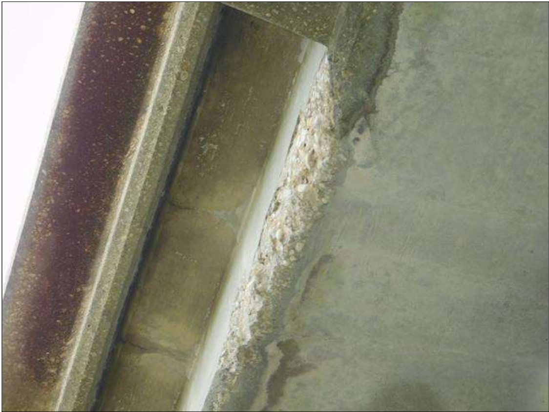
Span 2 Deck: SPALL LEFT OVERHANG 2 FEET X 6 INCH X 1 INCH DEEP
