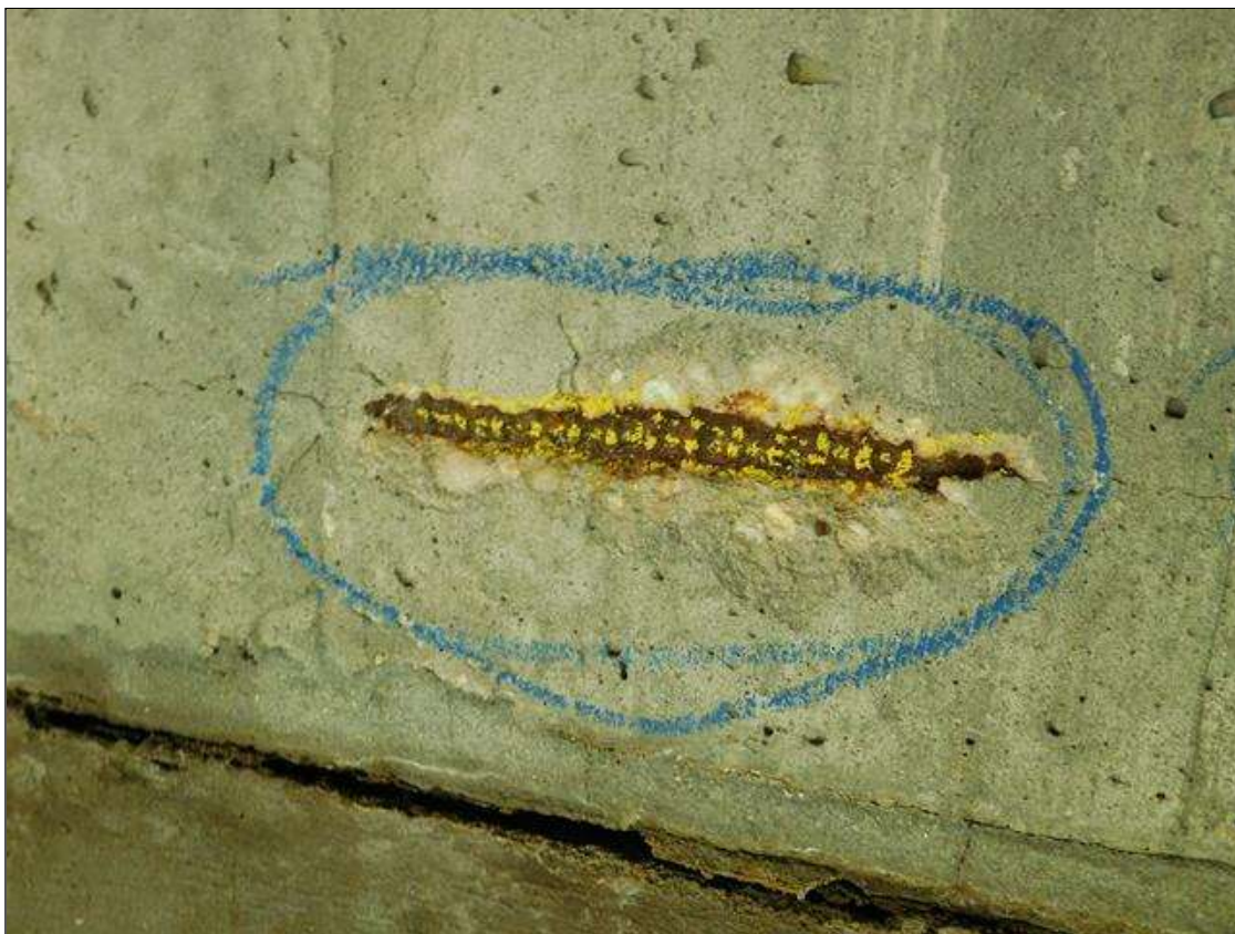
End Bent 2 Abutment: 1 FOOT OF EXPOSED REBAR IN BAY 2.
