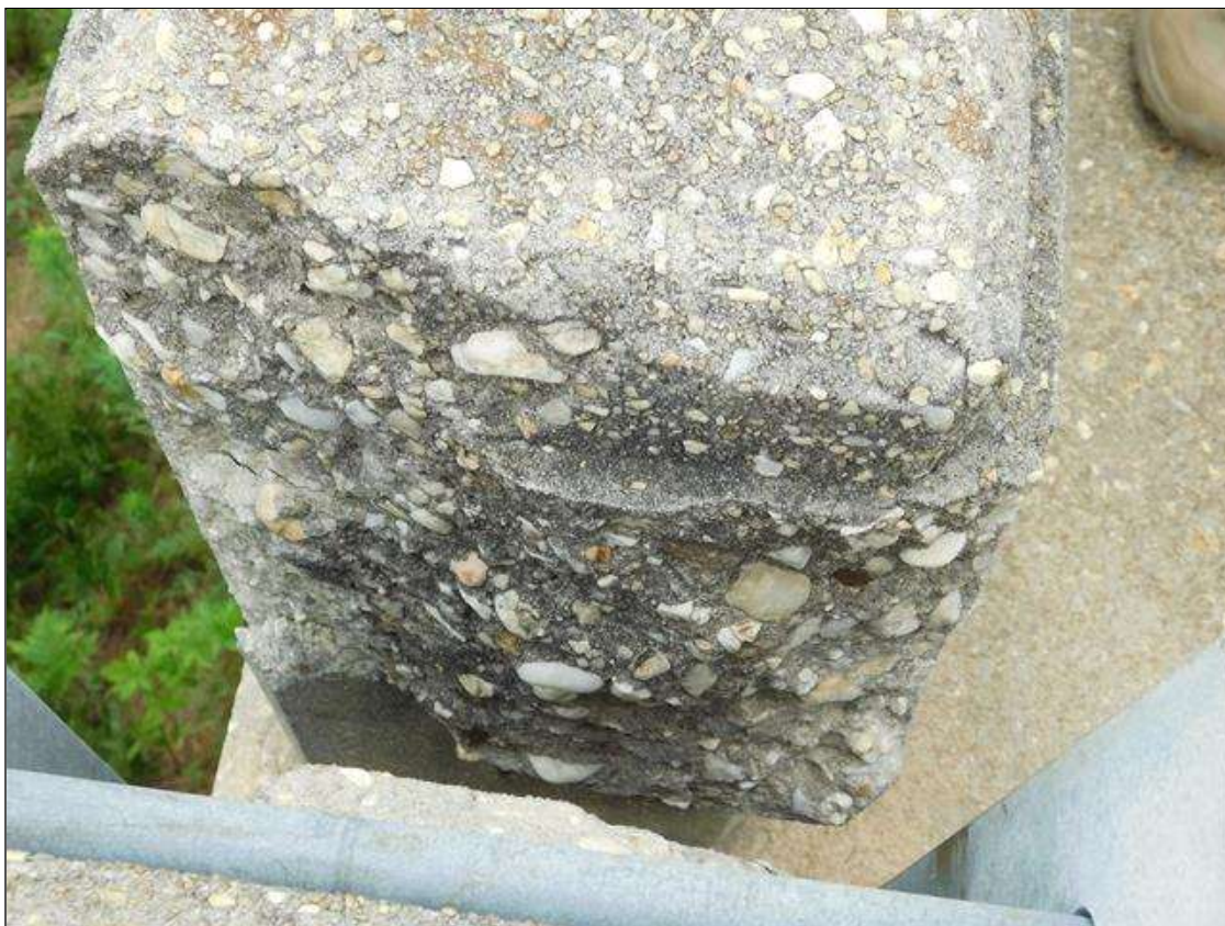
Span 4 Right Bridge Rail: 1 FOOT OF SPALLING WITH EXPOSED REBAR IN POST #6.
