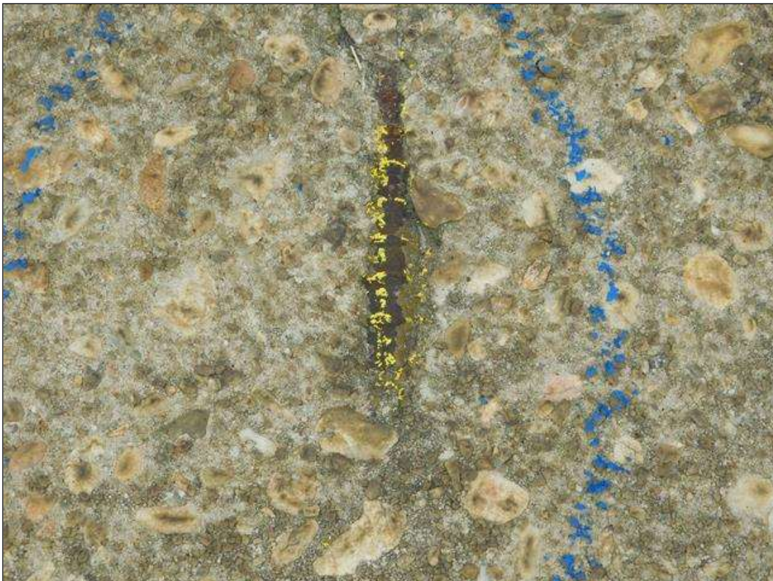
Span 3 Deck: 1 SQUARE FOOT OF EXPOSED REBAR IN THE LEFT CURB.
