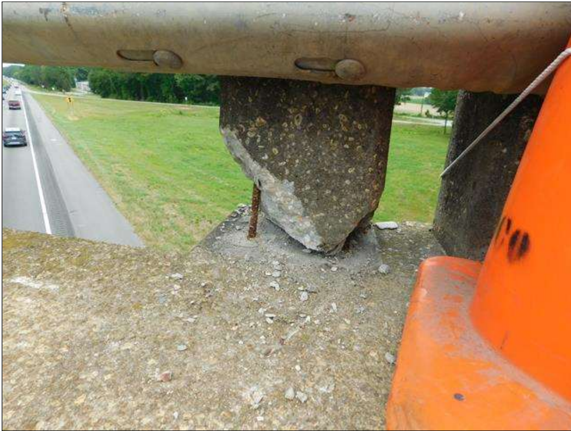
Span 2 Right Bridge Rail: IMPACT DAMAGE. THE 4TH GUARDRAIL POST FROM BENT 1 IS CRACKED, SPALLED AND LEANING OUT 1.5" AT TOP (REFERENCED FROM POST 3). HORIZONTAL RAILING FROM POST 4 TO POST 5 IS CRACKED AND PUSHED OUT. POSTS 5 & 6 HAVE WRAP-AROUND CRACKING AT BOTTOM OF POSTS BUT APPEAR TO BE PLUMB. TEMPORARY STEEL GUARDRAIL HAS BEEN ADDED FROM POST 3 TO POST 7. AFFECTED AREA IS OVER THE NORTHBOUND LANES OF I-95. PAR ISSUED.
