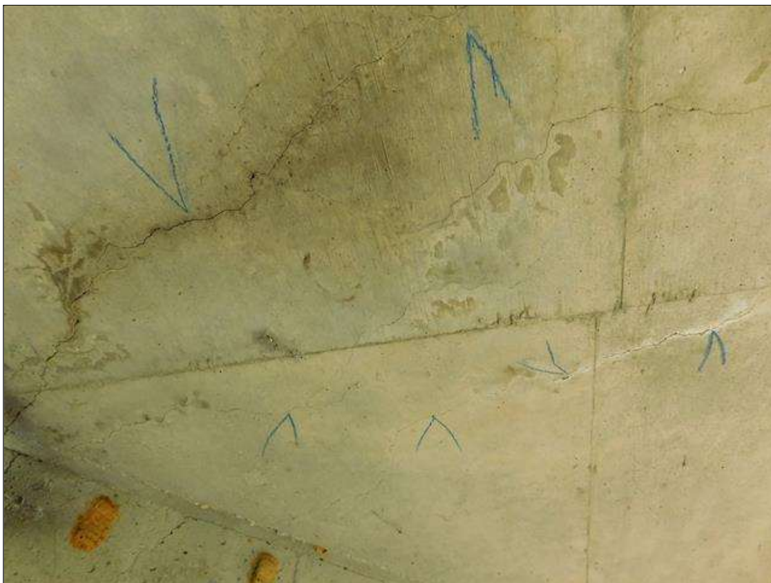
Span 4 Deck: 5 FEET OF 1/16 INCH TRANSVERSE AND MAP-CRACKING IN BOTTOM OF DECK BAY 3
