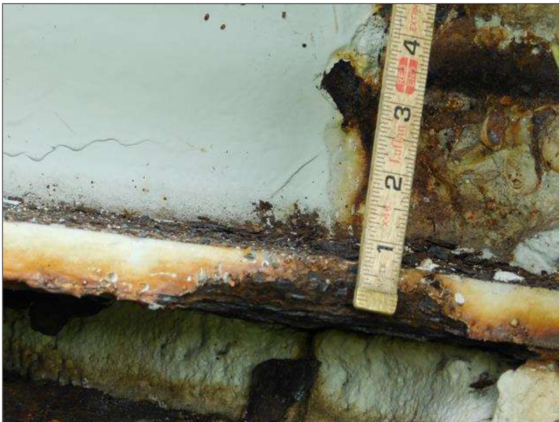
Span 1 Beam 1: 1/4" SECTION LOSS IN BOTTOM FLANGE BETWEEN BACKWALL AND NEAR BEARING ASSEMBLY (NOT IN BEARING AREA) WITH 3/4 INCH REMAINING AT END BENT 1.
