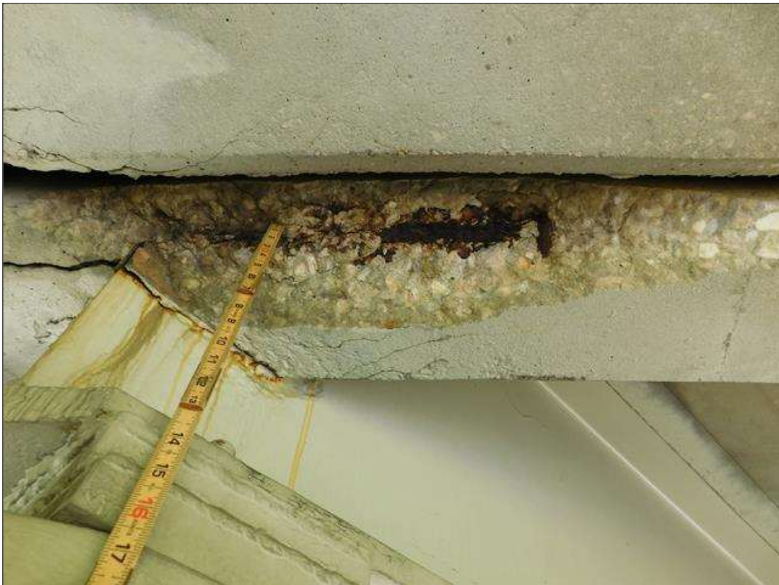
Span 3 Deck: 36" LONG SPALL 6" WIDE X 3" DEEP WITH SECTION LOSS TO EXPOSED REBAR (ESTIMATED 3/4" REMAINING) IN END DIAPHRAGM AT BENT 2 BAY 2. PAR ISSUED.
