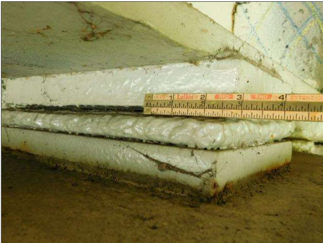
Span 4 Beam 3 - Far Bearing: SECTION LOSS ARRESTED. PITTED 1/8 INCH DEEP IN VERTICAL FACES. COATING GOOD. OTHER BEARING ASSEMBLIES SIMILAR THROUGHOUT STRUCTURE.
