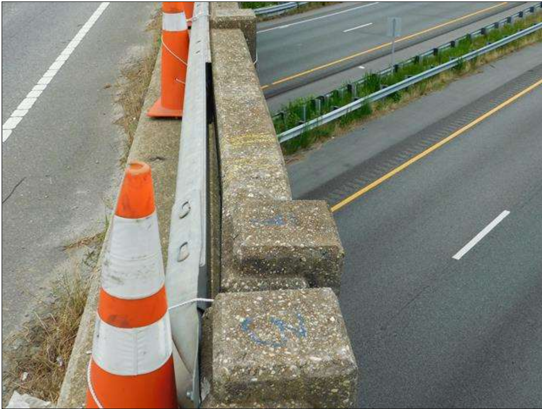
Span 2 Right Bridge Rail: IMPACT DAMAGE. THE 4TH GUARDRAIL POST FROM BENT 1 IS CRACKED, SPALLED AND LEANING OUT 1.5" AT TOP (REFERENCED FROM POST 3). HORIZONTAL RAILING FROM POST 4 TO POST 5 IS CRACKED AND PUSHED OUT. POSTS 5 & 6 HAVE WRAP-AROUND CRACKING AT BOTTOM OF POSTS BUT APPEAR TO BE PLUMB. TEMPORARY STEEL GUARDRAIL HAS BEEN ADDED FROM POST 3 TO POST 7. AFFECTED AREA IS OVER THE NORTHBOUND LANES OF I-95. PAR ISSUED.
