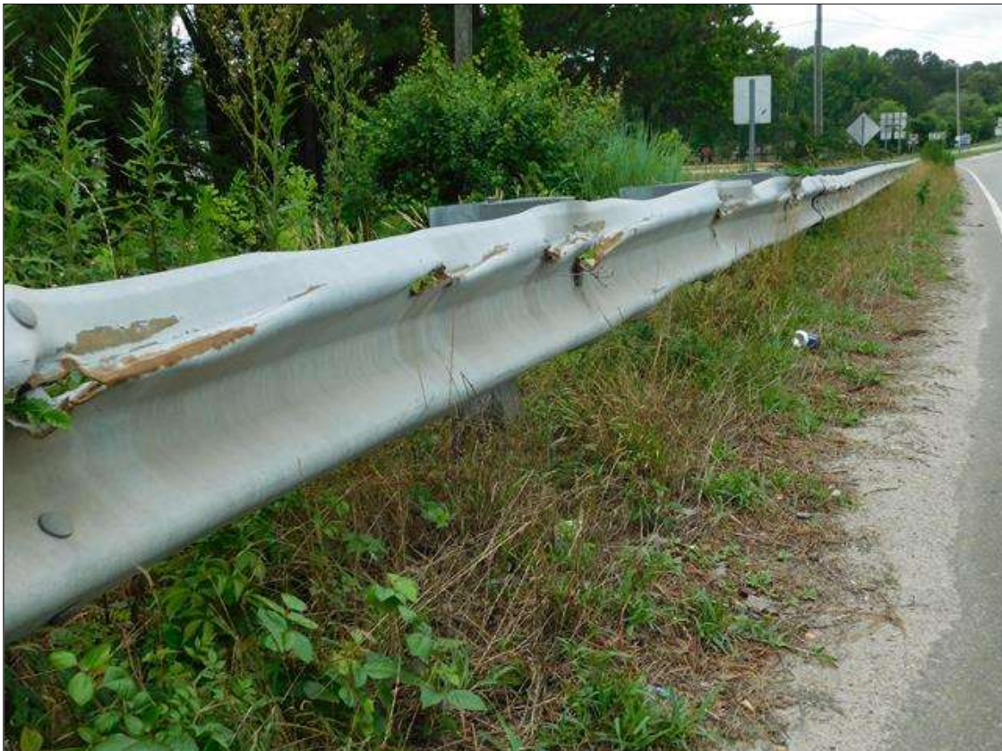
27 FEET OF IMPACT/SCRAPE DAMAGE ALONG THE LEFT SIDE APPROACH GUARDRAIL AT NORTH END WITH LOSS OF CONNECTION AT 4 POSTS. PAR ISSUED.
