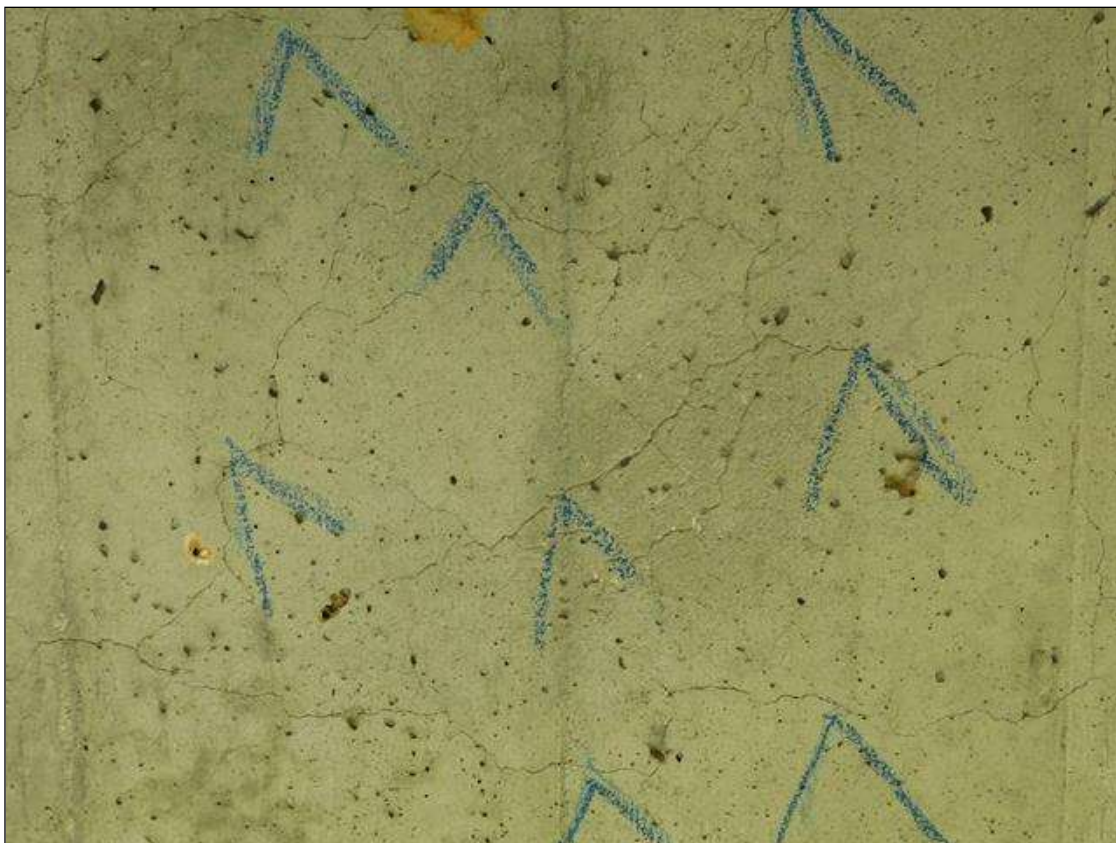
End Bent 2 Abutment: 28 FEET HAIRLINE MAP CRACKING FULL LENGTH
