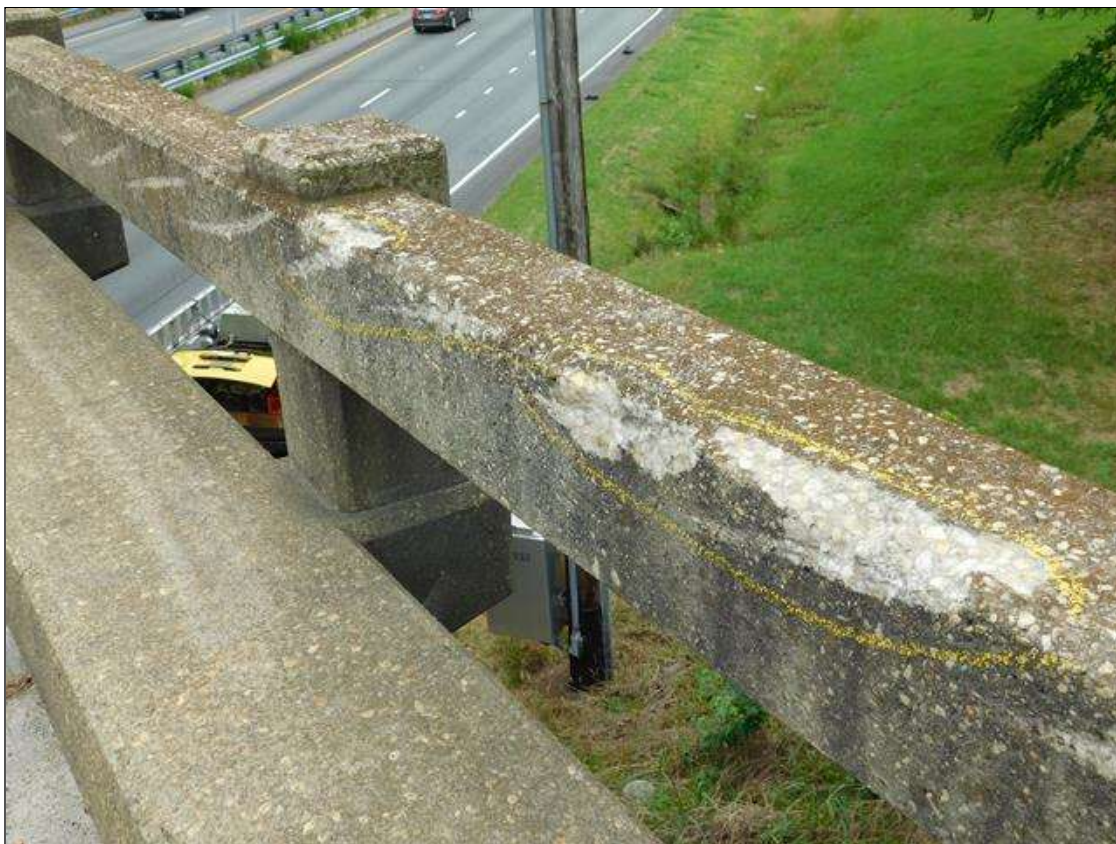
Span 4 Left Bridge Rail: 5 FEET OF IMPACT DAMAGE ALONG RAIL.
