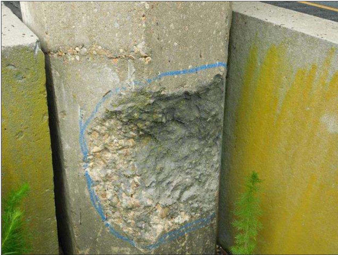
Bent 2 Pile 7: SPALL 1 FOOT FROM GROUNDLINE 4 INCH DEEP X 16 INCH DIAMETER RIGHT SIDE WITH 3 1/32 INCH HORIZONTAL CRACKS LEFT SIDE OPPOSITE SPALL
