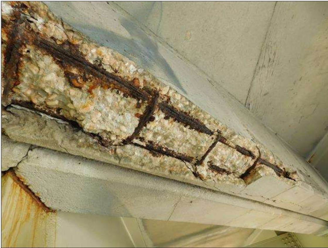
Span 3 Deck: 6' OF SPALLING AND DELAMINATION WITH SECTION LOSS TO EXPOSED REBAR (ESTIMATED 1 INCH REMAINING) 4 INCHES DEEP X 6 FEET LONG X 10 INCHES WIDE IN SPAN 3 END DIAPHRAGM OVER BENT 3, BAY 2. PAR ISSUED.
