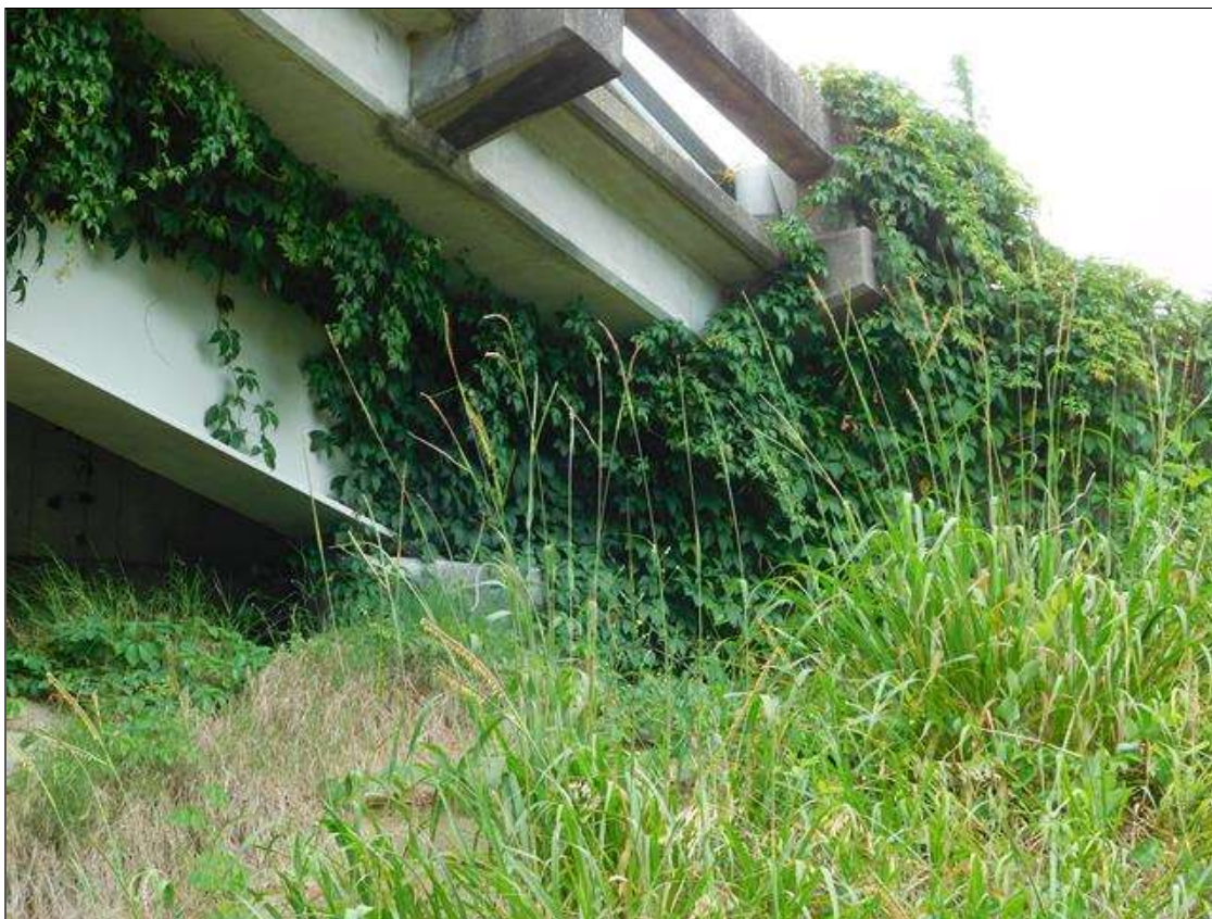
VEGETATION GROWTH AT ENDS OF BRIDGE
