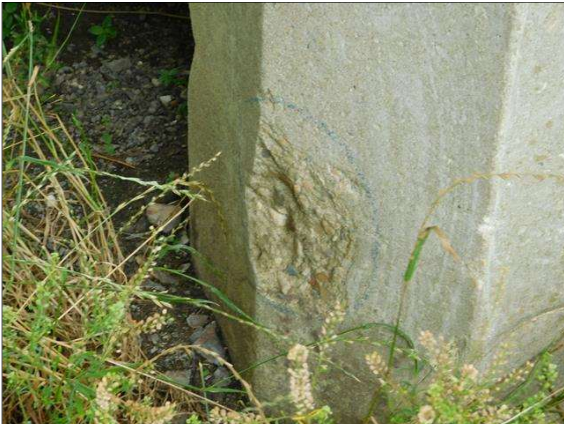
Bent 1 Pile 3: 5 INCH DIAMETER SPALL 1/2 INCH DEEP GROUNDLINE
