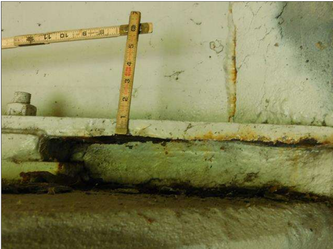
Span 1 Beam 4: 1/8" SECTION LOSS IN THE BOTTOM FLANGE AT END BENT 1 WITH 7/8 INCH REMAINING BETWEEN BACKWALL AND BEARING ASSEMBLY (NOT IN BEARING AREA)
