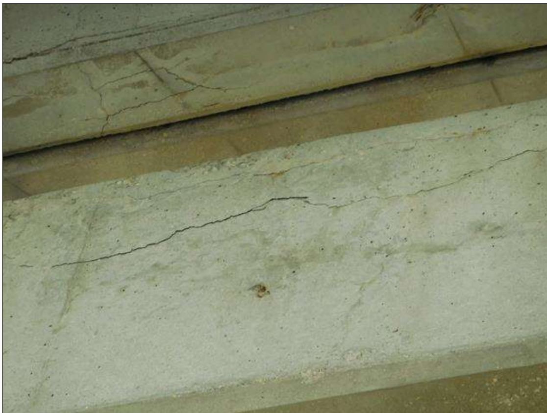
Bent 3 Cap 1: DELAMINATION IN FACE OF CAP SPAN 3 SIDE UNDER BAY 1.
