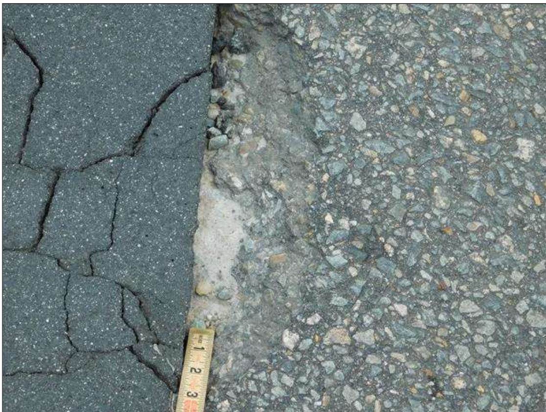
Span 1 Wearing Surface: 1 SQUARE FOOT FULL DEPTH POTHOLE IN THE SOUTHBOUND LANE AT BENT 1.
