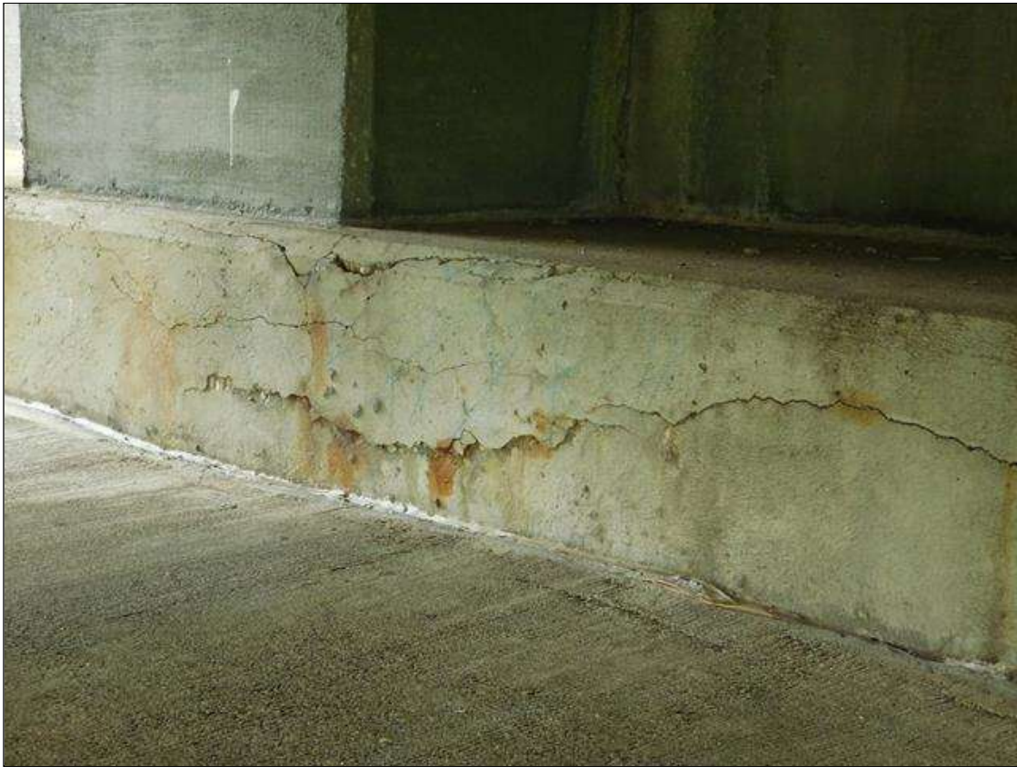
End Bent 2 Cap 1: 8 FEET LONGITUDINAL CRACKING FACE AND TOP WITH DELAMINATION AND RUST STAINING IN BAY 1.
