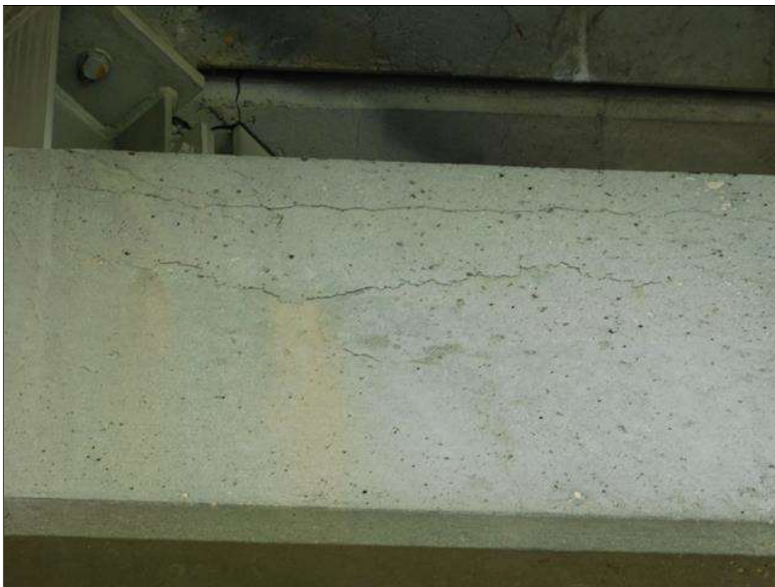
Bent 3 Cap 1: 3 FEET 1/8 INCH LONGITUDINAL IN FACE OF CAP SPAN 3 SIDE BEAM 3
