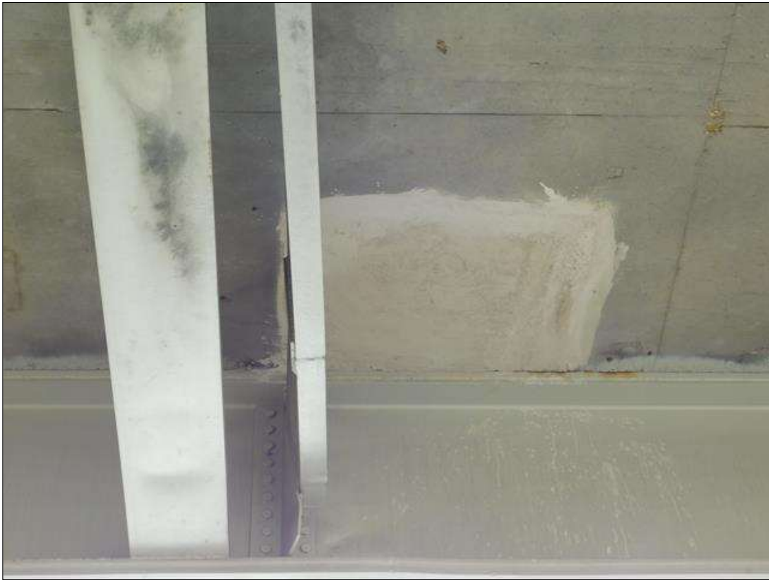
Span 2 Deck: 10 SQUARE FEET OF SOUND PATCHING IN BOTTOM OF DECK BAY 1 AT 1/3 POINT FROM BENT 1. THIS AREA WAS PREVIOUSLY DELAMINATING OVER LANES OF TRAFFIC AND WAS ISSUED A PRIORITY MAINTENANCE AND HAS BEEN REPAIRED SINCE LAST INSPECTION.
