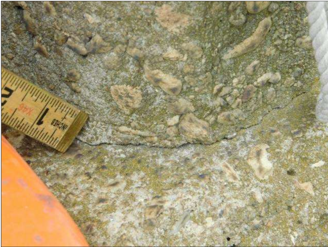
Span 2 Right Bridge Rail: IMPACT DAMAGE. THE 4TH GUARDRAIL POST FROM BENT 1 IS CRACKED, SPALLED AND LEANING OUT 1.5" AT TOP (REFERENCED FROM POST 3). HORIZONTAL RAILING FROM POST 4 TO POST 5 IS CRACKED AND PUSHED OUT. POSTS 5 & 6 HAVE WRAP-AROUND CRACKING AT BOTTOM OF POSTS BUT APPEAR TO BE PLUMB. TEMPORARY STEEL GUARDRAIL HAS BEEN ADDED FROM POST 3 TO POST 7. AFFECTED AREA IS OVER THE NORTHBOUND LANES OF I-95. PAR ISSUED.
