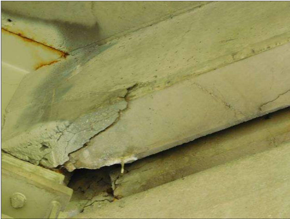
Span 1 Deck: BOTTOM OF DECK: 1/4 INCH WIDE CRACK LEFT OVERHANG DIAPHRAGM. CRACKING IN BAY 1, 2 AND 3 DIAPHRAGMS.
