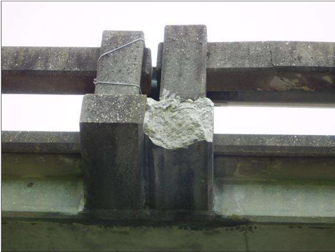
Span 2 Right Bridge Rail: IMPACT DAMAGE. THE 4TH GUARDRAIL POST FROM BENT 1 IS CRACKED, SPALLED AND LEANING OUT 1.5" AT TOP (REFERENCED FROM POST 3). HORIZONTAL RAILING FROM POST 4 TO POST 5 IS CRACKED AND PUSHED OUT. POSTS 5 & 6 HAVE WRAP-AROUND CRACKING AT BOTTOM OF POSTS BUT APPEAR TO BE PLUMB. TEMPORARY STEEL GUARDRAIL HAS BEEN ADDED FROM POST 3 TO POST 7. AFFECTED AREA IS OVER THE NORTHBOUND LANES OF I-95. PAR ISSUED.
