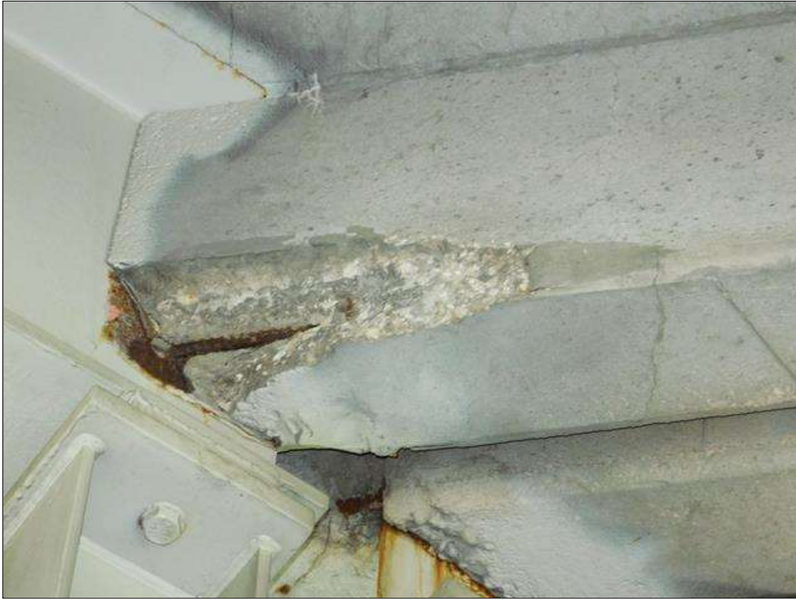
Span 2 Deck: 12 INCH X 8 INCH X 3 INCH DEEP SPALL WITH EXPOSED REBAR (WITHOUT SECTION LOSS) IN END DIAPHRAGM AT BENT 1 BAY 2.
