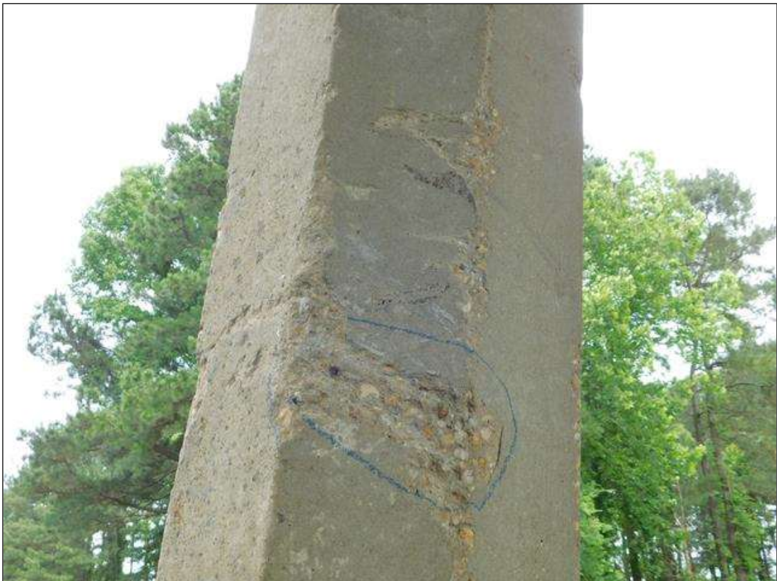
Bent 2 Pile 1: 1 FOOT SPALLING 1 INCH DEEP SPAN 2 SIDE
