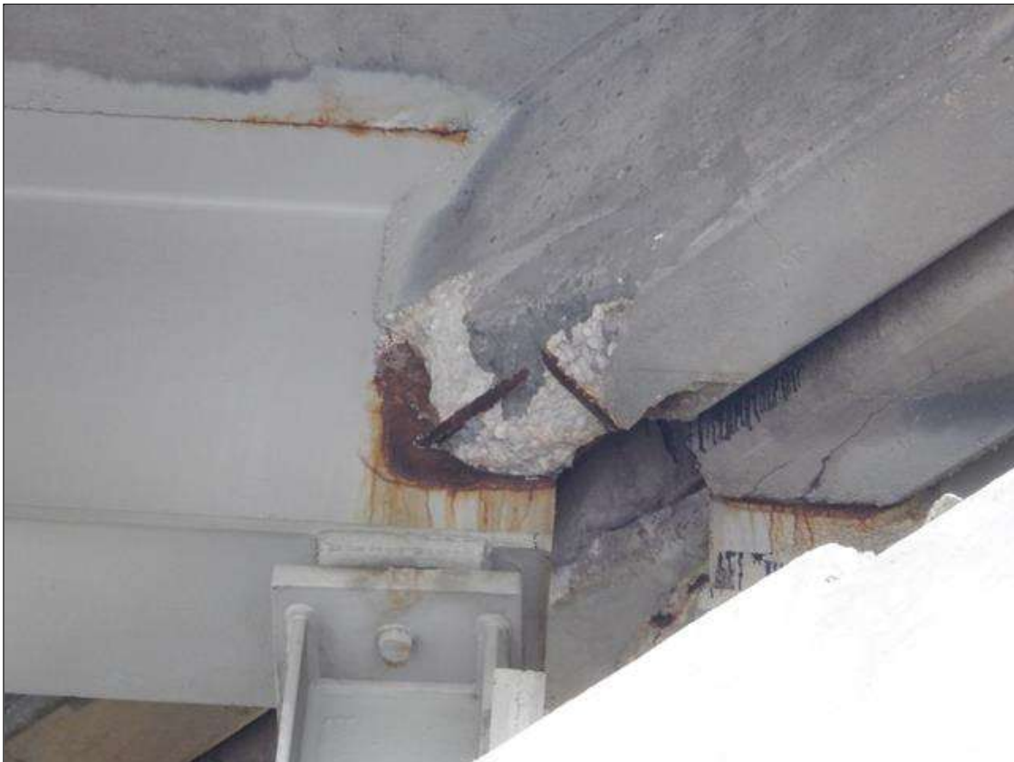
Span 2 Deck: PAR. BAY 1 NEAR DIAPHRAGM ADJACENT TO BEAM 2 SPALL WITH EXPOSED REBAR 1 FOOT X 4 INCHES X 4 INCHES, 5 PERCENT SECTION LOSS.
