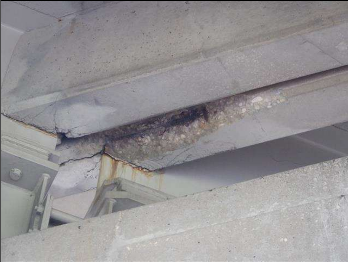
Span 3 Deck: PAR. 36 INCHES LONG SPALL 6 INCHES WIDE X 3 INCHES DEEP WITH SECTION LOSS TO EXPOSED REBAR (ESTIMATED 3/4 INCH REMAINING) IN END DIAPHRAGM AT BENT 2 BAY 2.
