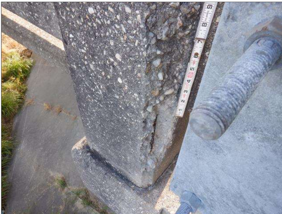
Span 1 Left Bridge Rail: 1 FOOT OF SPALLING IN POST 3 WITH EXPOSED REBAR, NO SECTION LOSS.
