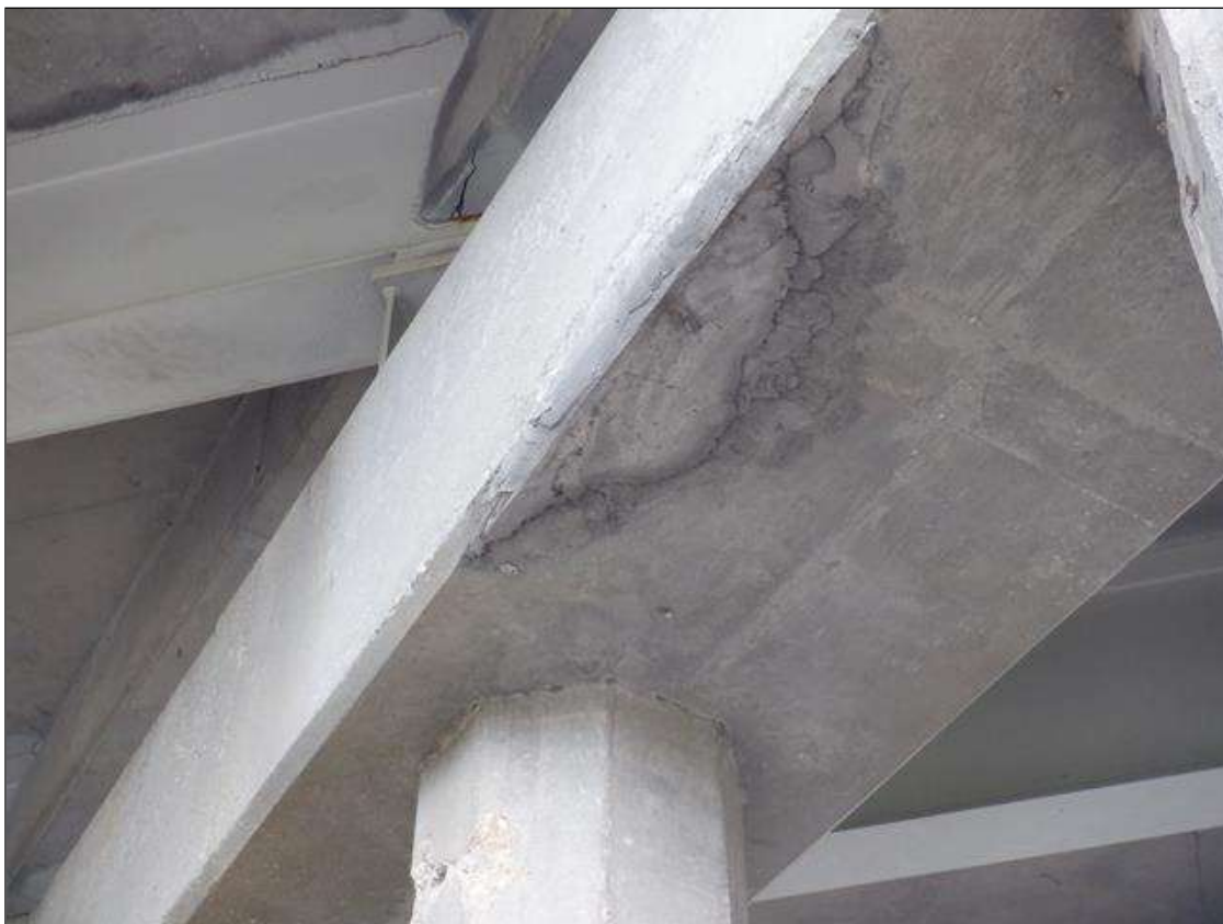
Bent 2 Cap 1: 3 FEET OF UNSOUND PATCHING BOTTOM OF CAP BAY 3
