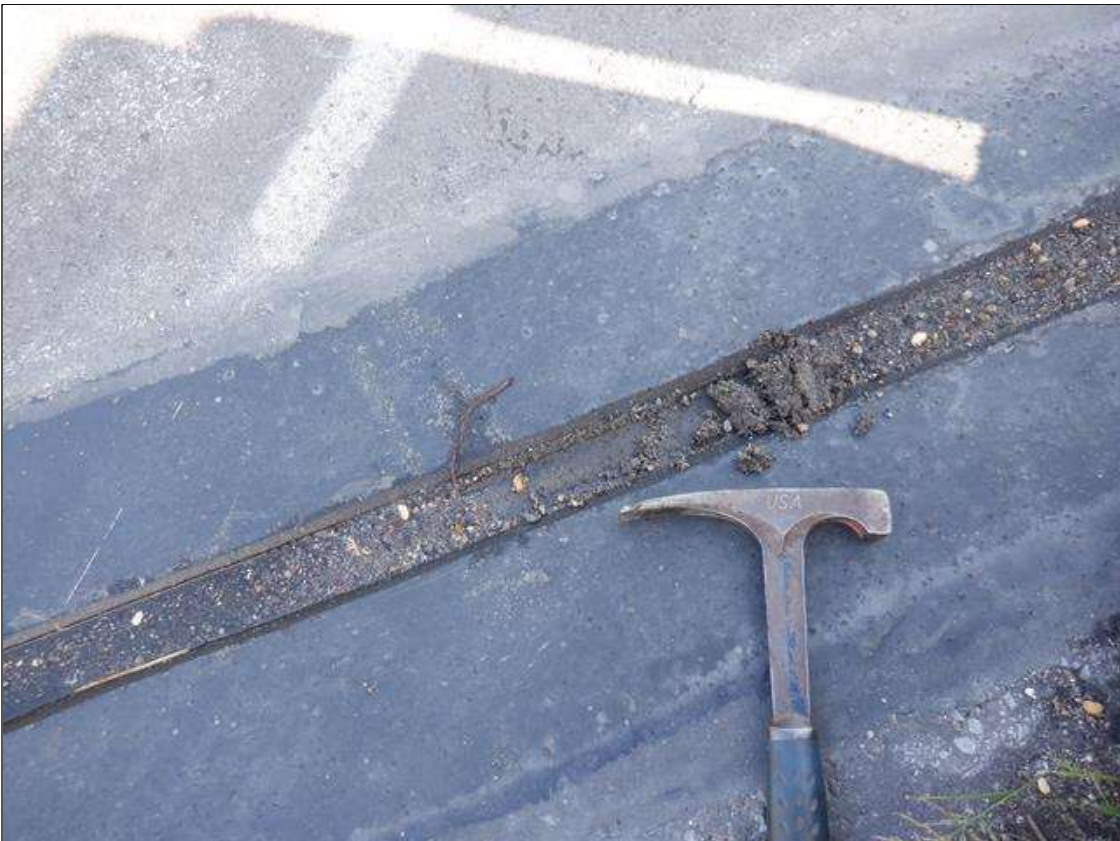
Span 3 Expansion Joint 3: IN BOTH SHOULDERS 2 FEET DIRT AND DEBRIS IMPACTION. STILL ALLOWS FREE JOINT MOVEMENT.
