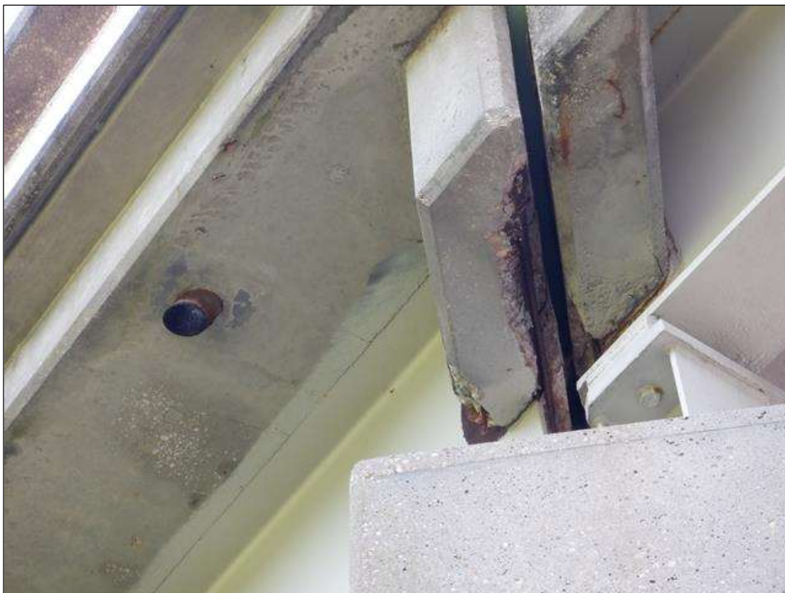
Span 1 Deck: PAR. RIGHT OVERHANG DIAPHRAGM SPALL WITH EXPOSED REBAR 2 FEET X 5 INCHES X UP TO 1 FOOT, 5 PERCENT SECTION LOSS.
