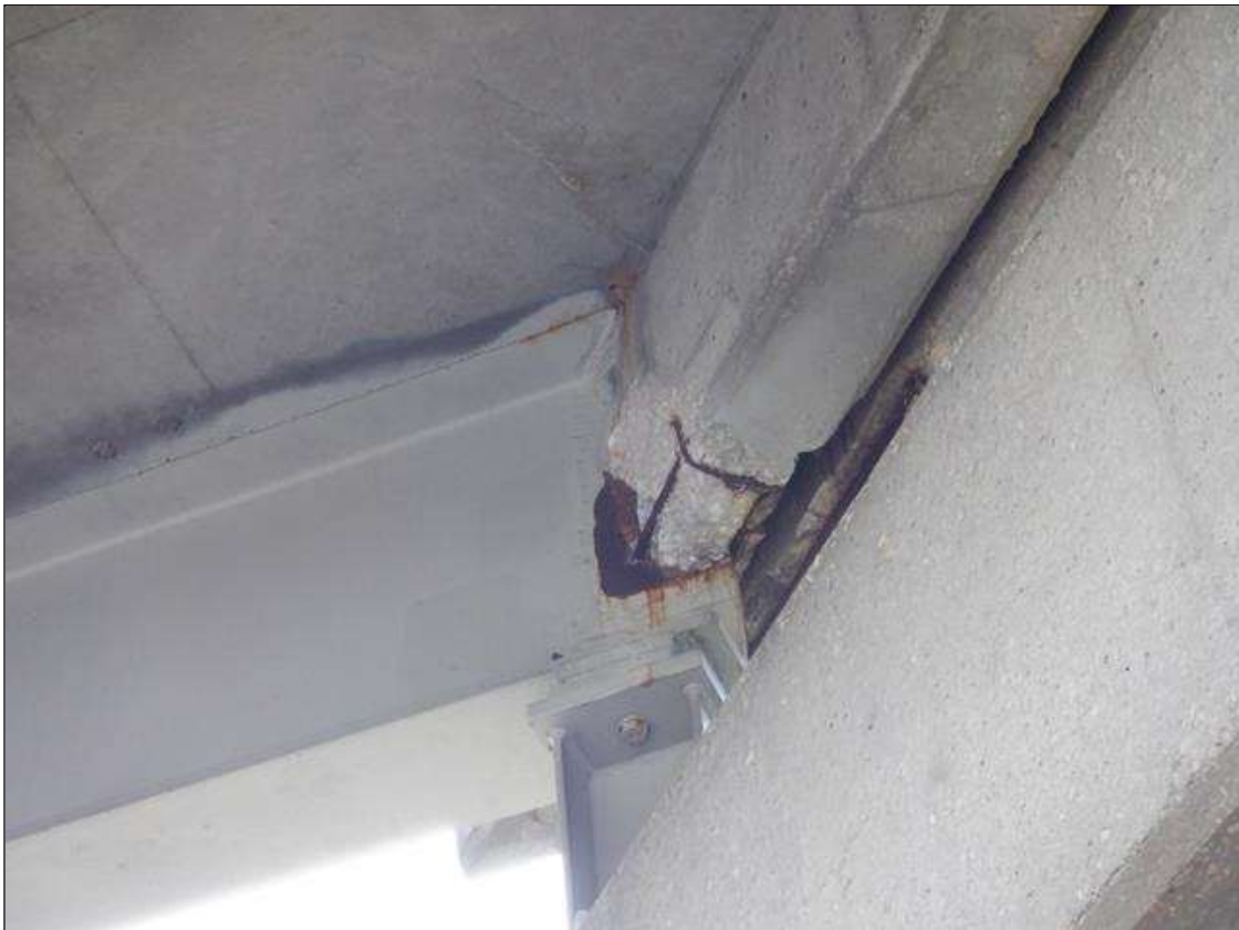
Span 2 Deck: PAR. BAY 3 DIAPHRAGM OVER BENT 1 ADJACENT TO BEAM 4 SPALL WITH EXPOSED REBAR 1 FOOT X 8 INCHES X 3 INCHES DEEP. 5 PERCENT SECTION LOSS.
