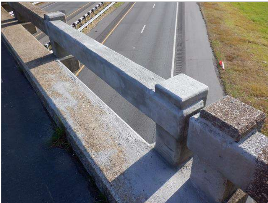
Span 2 Right Bridge Rail: PREVIOUS IMPACT DAMAGE FROM POST 3 TO 5 HAS BEEN REPAIRED.
