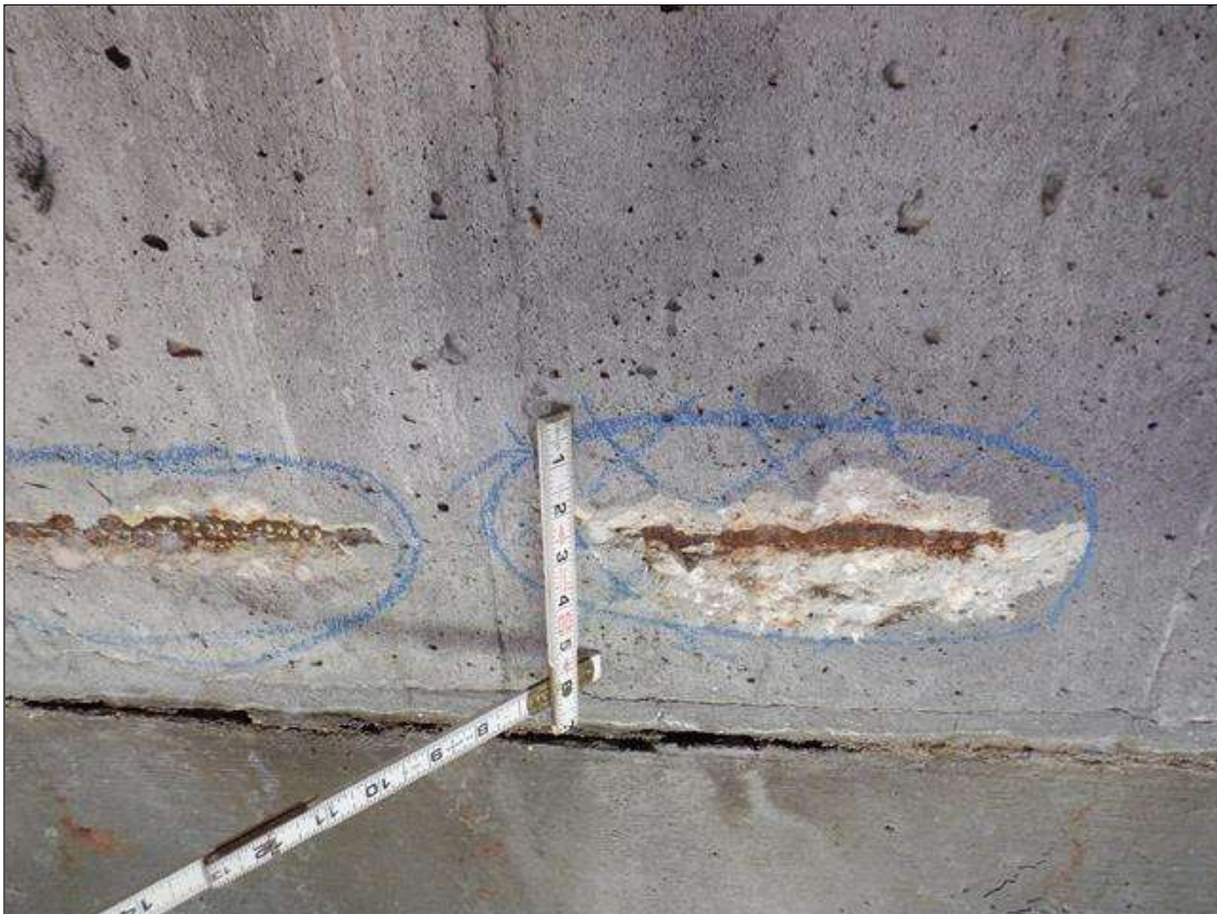
End Bent 2 Abutment: SPALL WITH EXPOSED REBAR IN BAY 2 ADJACENT TO EXPOSED REBAR. 1 FOOT X 5 INCHES, NO SECTION LOSS.
