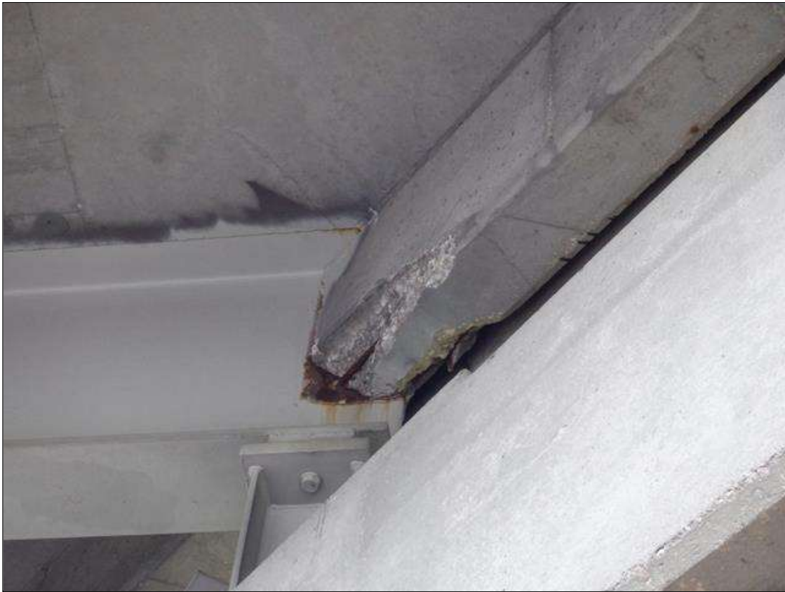
Span 2 Deck: 12 INCHES X 8 INCHES X 3 INCHES DEEP SPALL WITH EXPOSED REBAR (WITHOUT SECTION LOSS) IN END DIAPHRAGM AT BENT 1 BAY 2.
