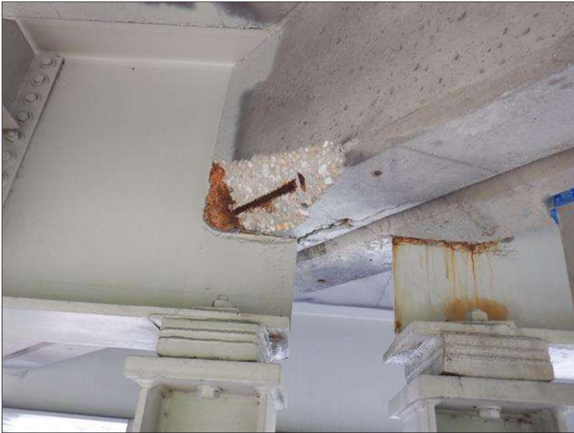
Span 4 Deck: PAR. BAY 2 DIAPHRAGM ADJACENT TO BEAM 3 SPALL WITH EXPOSED REBAR 1 FOOT X 4 INCHES X 4 INCHES. 5 PERCENT SECTION LOSS.
