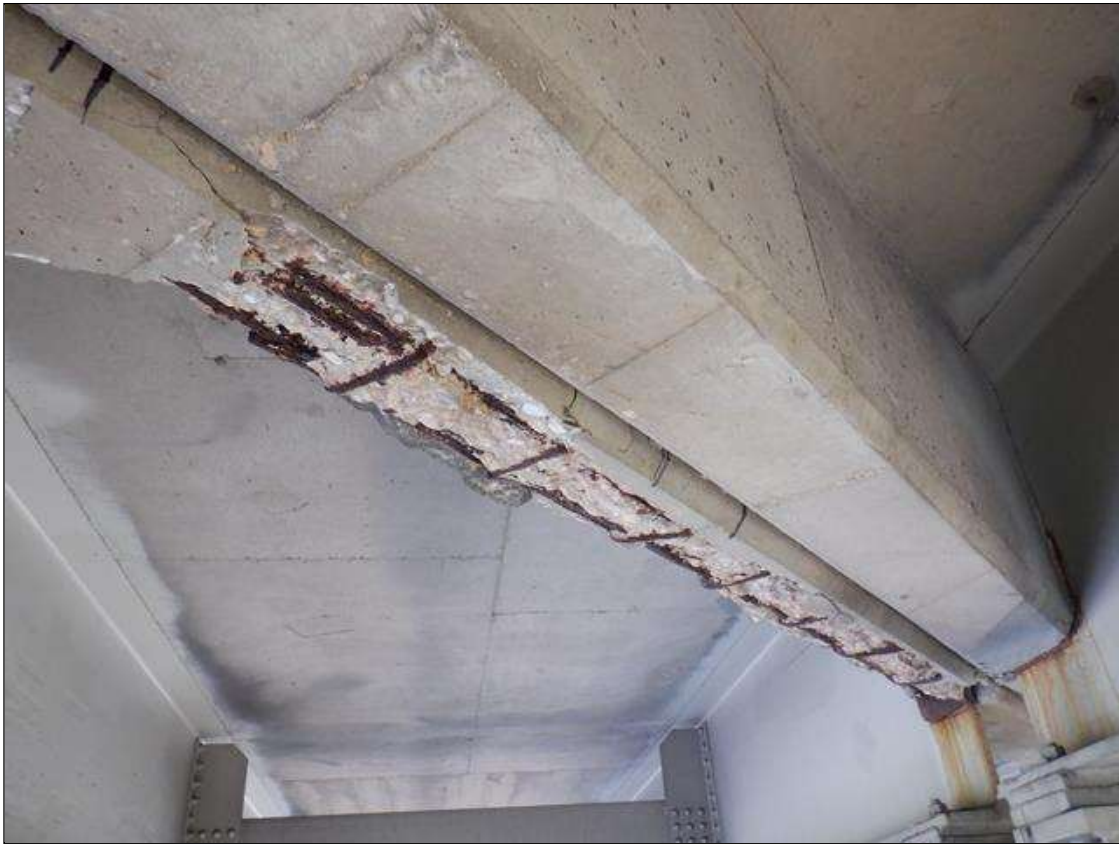
Span 3 Deck: PAR. 6 FEET OF SPALLING AND DELAMINATION WITH SECTION LOSS TO EXPOSED REBAR (ESTIMATED 1 INCH REMAINING) 4 INCHES DEEP X 6 FEET LONG X 10 INCHES WIDE IN SPAN 3 END DIAPHRAGM OVER BENT 3, BAY 2.
