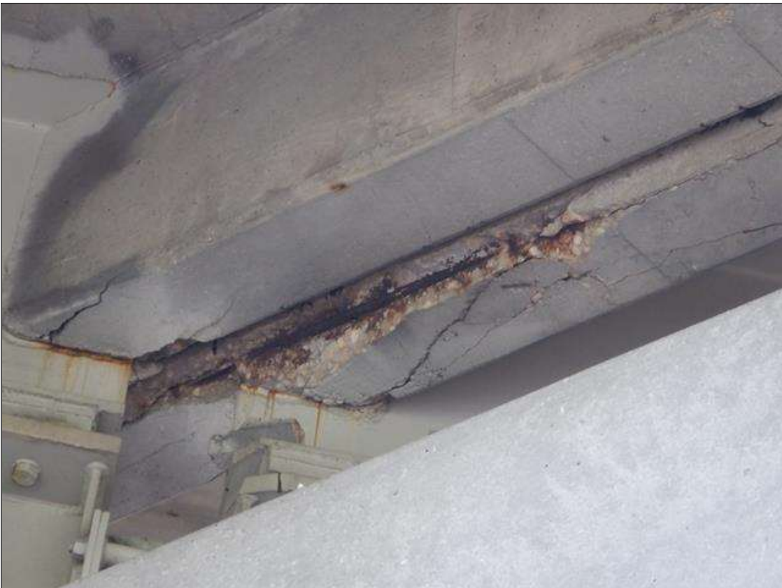
Span 3 Deck: PAR. BAY 3 DIAPHRAGM ADJACENT TO BEAM 3 SPALL WITH EXPOSED REBAR 4 FEET X 6 INCHES X 6 INCHES, 10 PERCENT SECTION LOSS.
