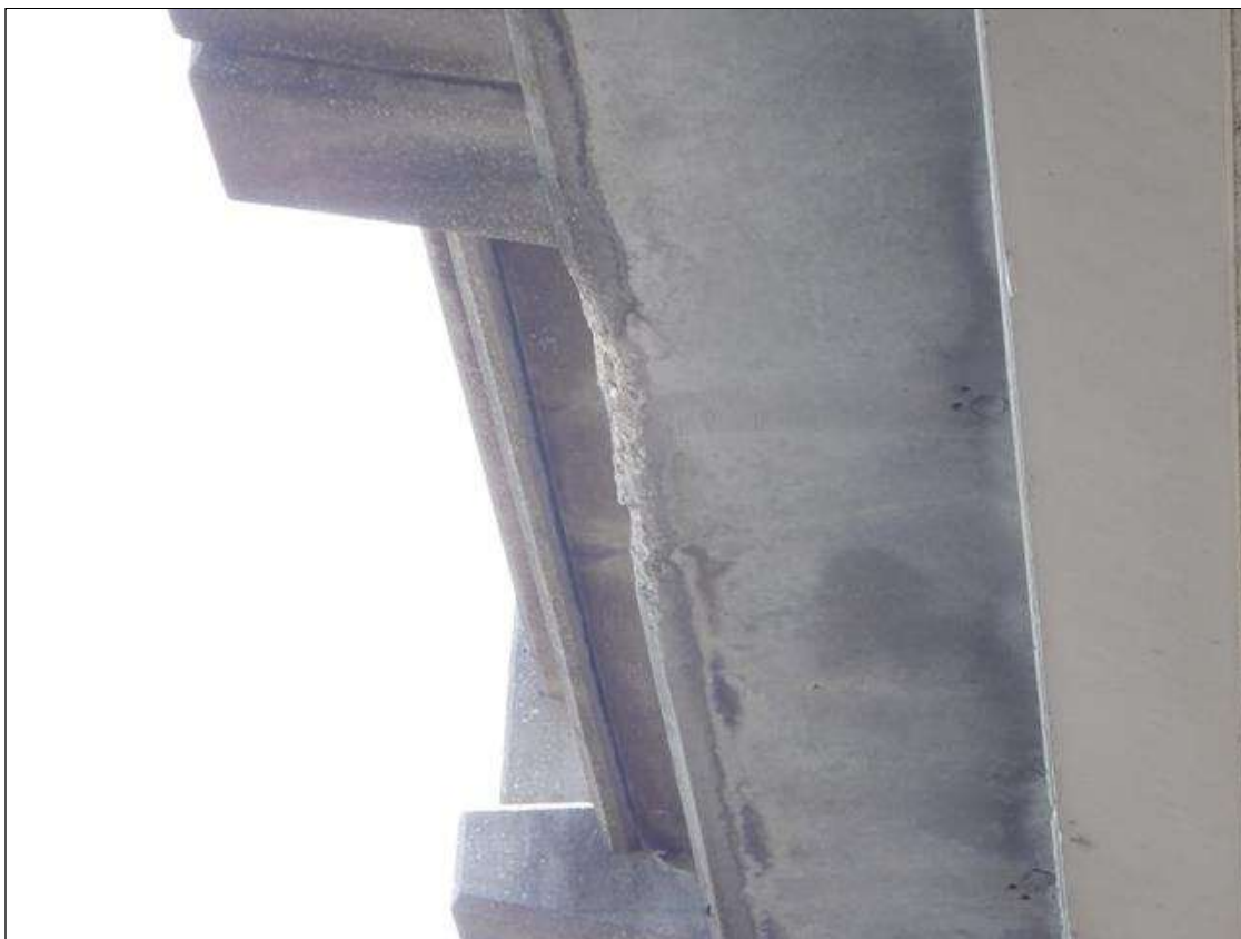
Span 2 Deck: BETWEEN RAIL POSTS 4 AND 5 AT LEFT OVERHANG CORNER 3 FEET X 2 INCHES X 2 INCHES SPALLING.
