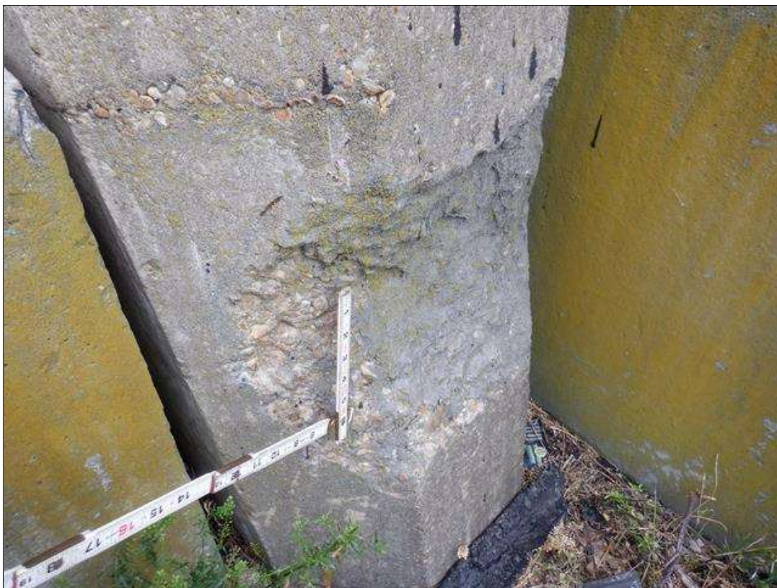
Bent 2 Pile 7: SPALL 1 FOOT FROM GROUNDLINE 4 INCHES DEEP X 16 INCHES DIAMETER RIGHT SIDE WITH THREE (3) 1/32 INCH HORIZONTAL CRACKS LEFT SIDE OPPOSITE SPALL.
