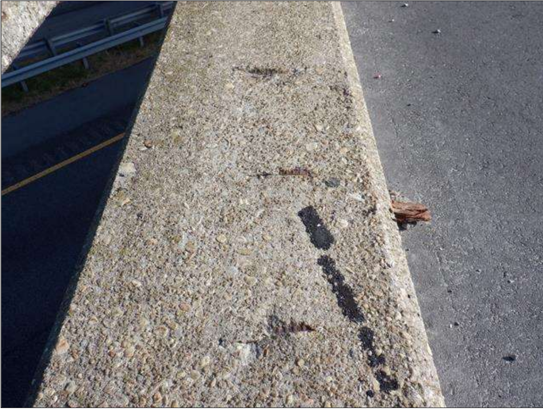
Span 2 Left Bridge Rail: ON TOP OF CURB SCATTERED THROUGHOUT 11 SPALLS WITH EXPOSED REBAR 2 INCHES X 3 INCHES X 1/4 INCH DEEP, NO SECTION LOSS
