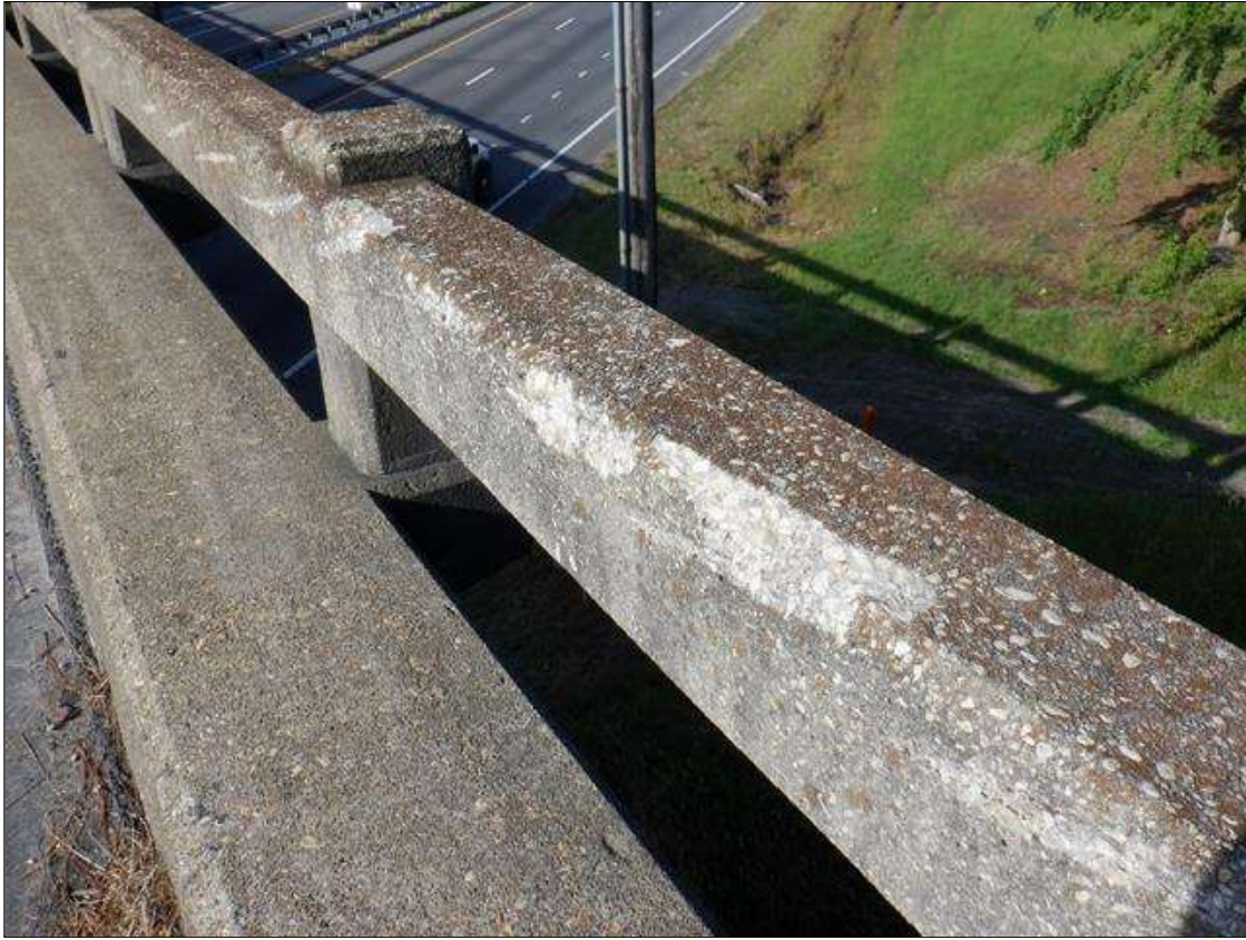
Span 4 Left Bridge Rail: 10 FEET OF IMPACT DAMAGE ALONG RAIL WITH SPALLS UP TO 1 FOOT X 2 INCHES X 2 INCHES.
