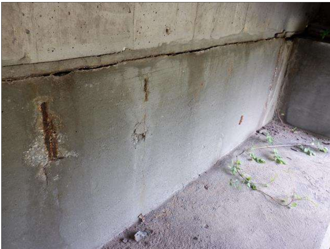
End Bent 2 Abutment: IN BAYS 2 AND 3, SPALLS WITH EXPOSED REBAR 6 INCHES X UP TO 18 INCHES X UP TO 1/4 INCH DEEP. NO SECTION LOSS.
