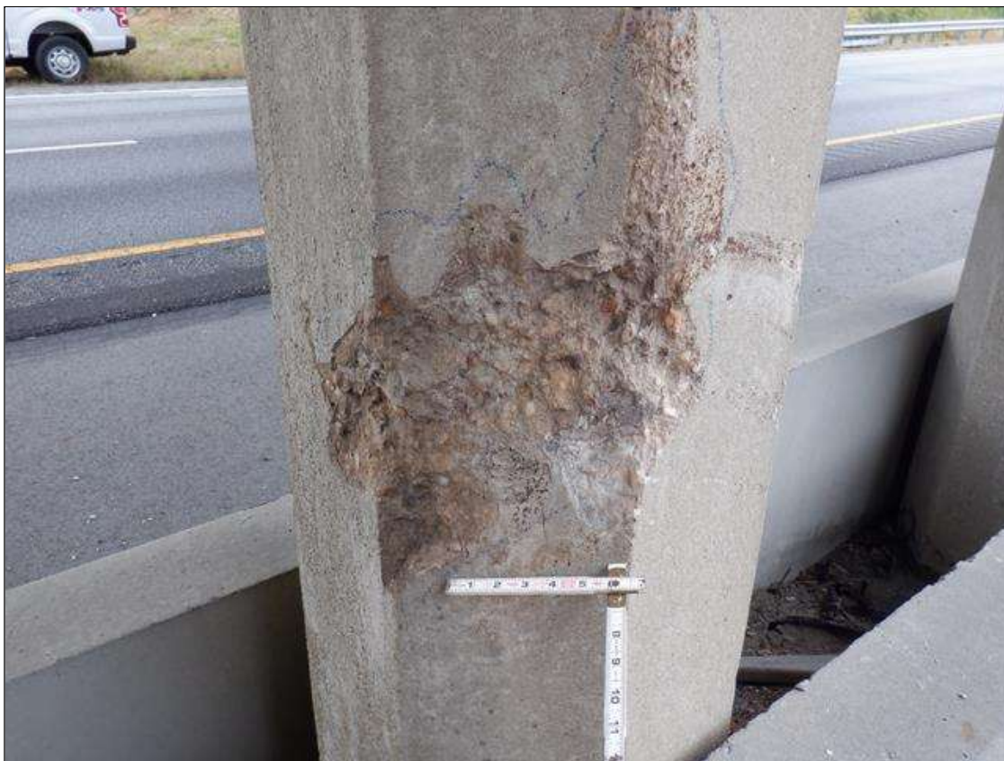
Bent 2 Pile 5: 5 SPALLS 1 INCH DEEP TOTALLING 6 SQUARE FEET
