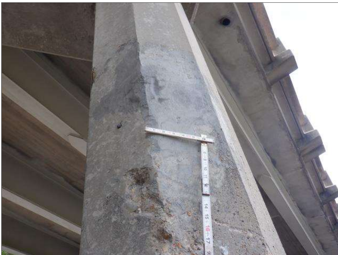
Bent 2 Pile 7: 2 FEET OF SOUND PATCHING SPAN 2 SIDE
