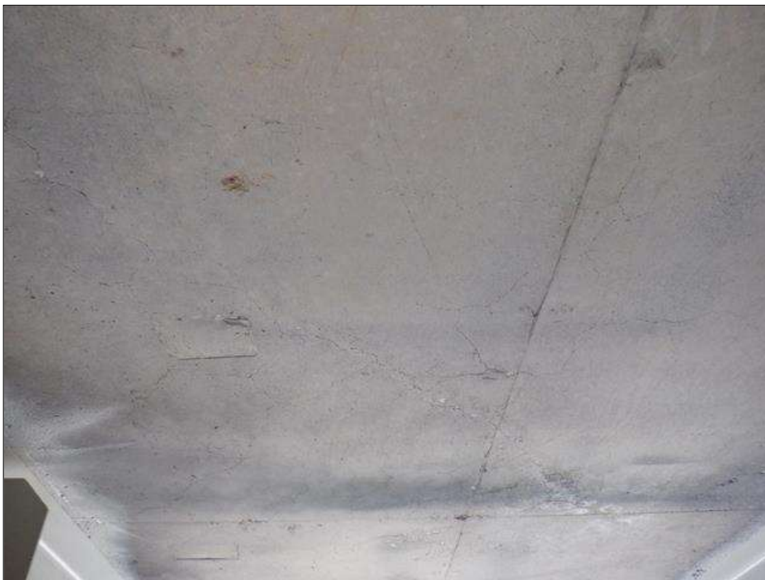
Span 1 Deck: BOTTOM OF DECK: HAIRLINE MAP TRANSVERSE AND DIAGONAL CRACKING IN ALL BAYS
