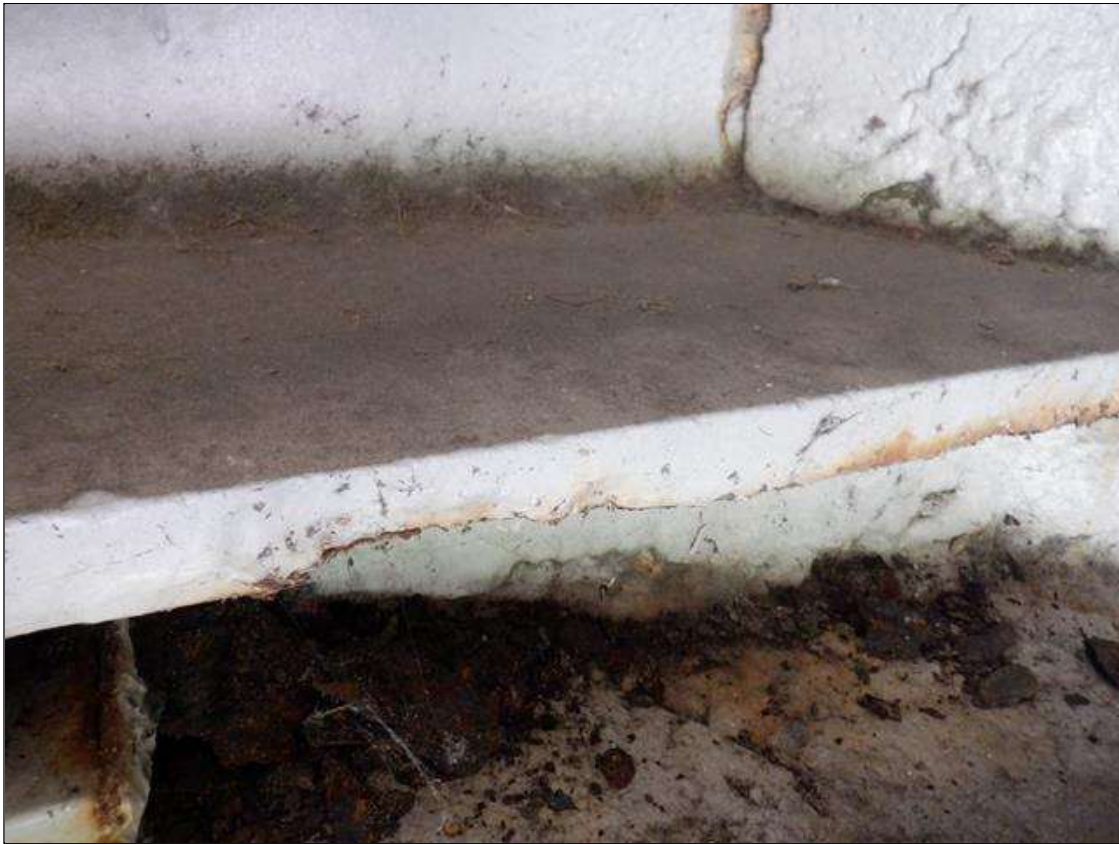
Span 1 Beam 1: 1/4 INCH SECTION LOSS IN BOTTOM FLANGE BETWEEN BACKWALL AND NEAR BEARING ASSEMBLY (NOT IN BEARING AREA) WITH 3/4 INCH REMAINING AT END BENT 1. SURFACE RUST IN WEB ADJACENT TO BACKWALL.
