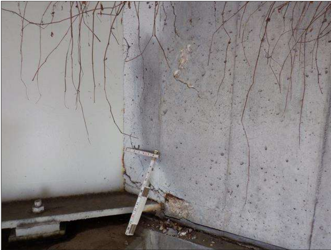
End Bent 1 Abutment: LEFT SIDE BEAM 2 BAY 1 DELAMINATION WITH SPALL AND EXPOSED REBAR. 2 FEET X 3 FEET X UP TO 1 INCH DEEP. NO SECTION LOSS.
