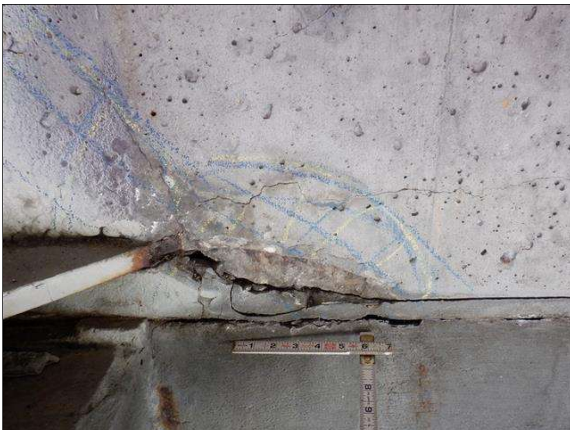
End Bent 2 Abutment: ADJACENT TO BEAM 3 IN BAY 3 SPALL 1 FOOT X 2 INCHES X UP TO 1 INCH DEEP.
