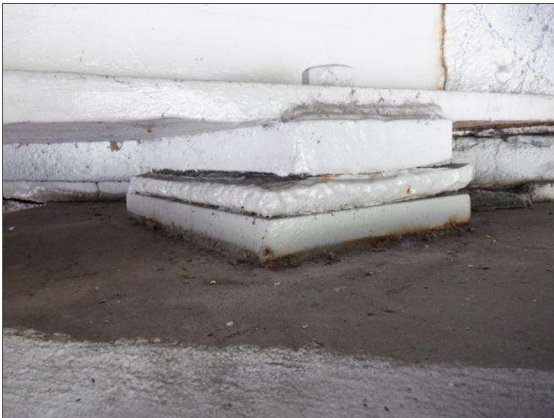
Span 4 Beam 3 - Far Bearing: SECTION LOSS ARRESTED. PITTED 1/8 INCH DEEP IN VERTICAL FACES. COATING GOOD.
