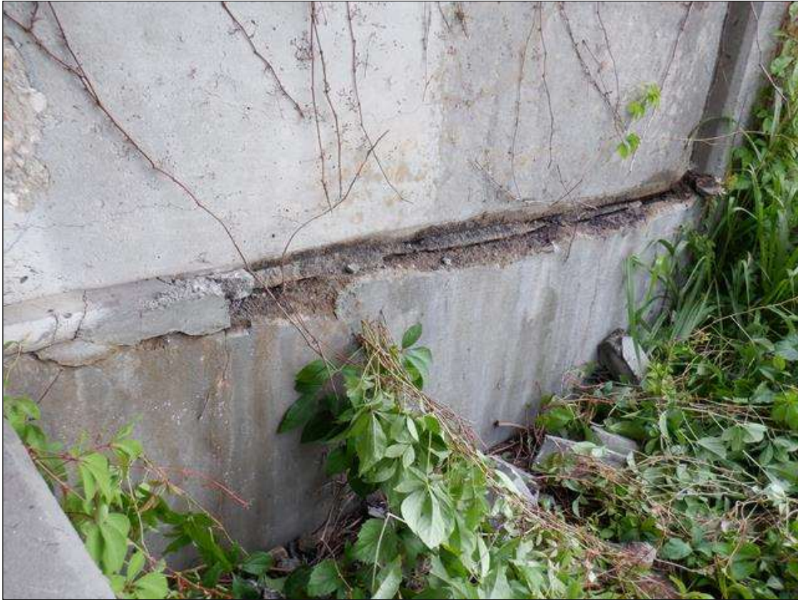
End Bent 1 Abutment: FROM LEFT END TO BEAM 1 CONCRETE IN JOINT SPALLED OFF 7 FEET X 4 INCHES X 4 INCHES.
