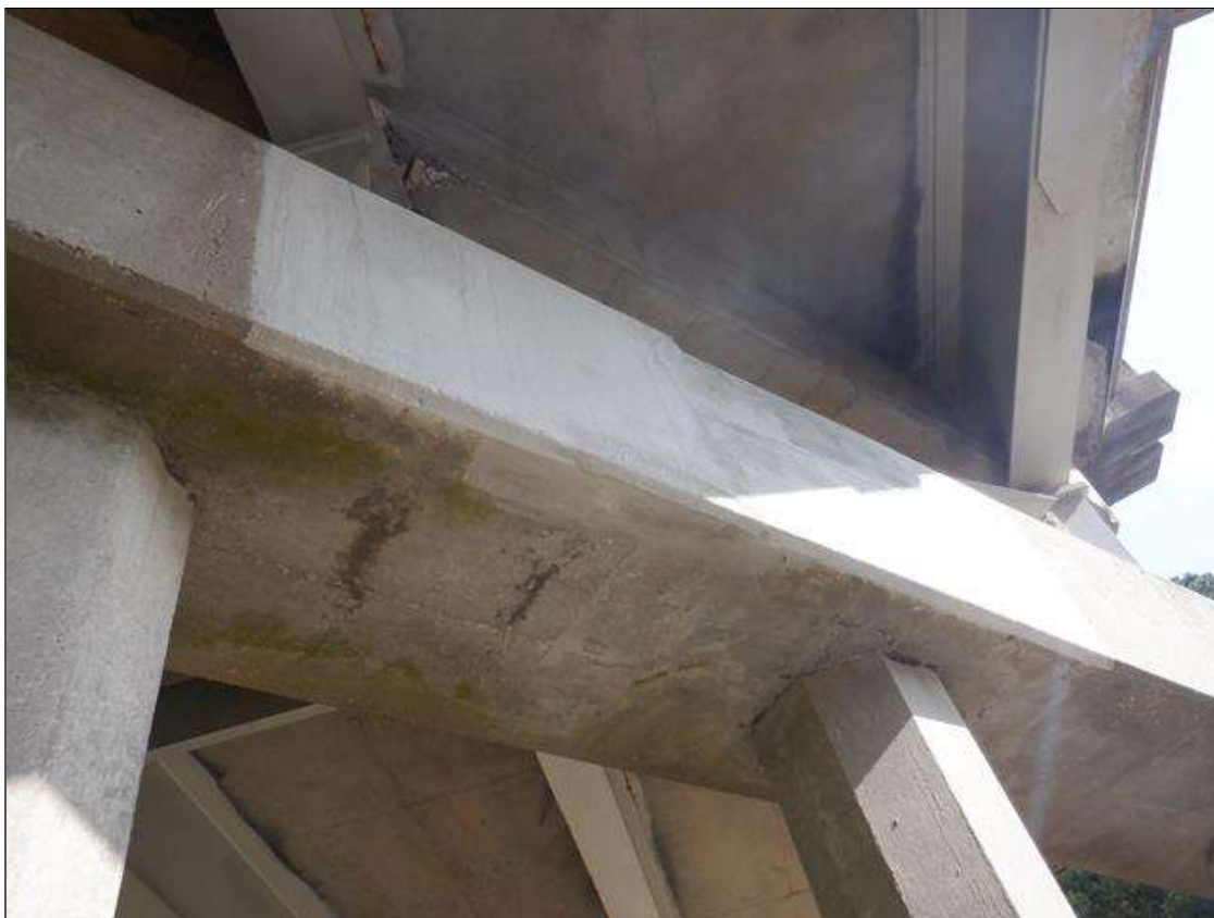
Bent 1 Cap 1: SPAN 2 SIDE UNDER BAY 1, 8 FEET X FULL HEIGHT SOUND PATCH.
