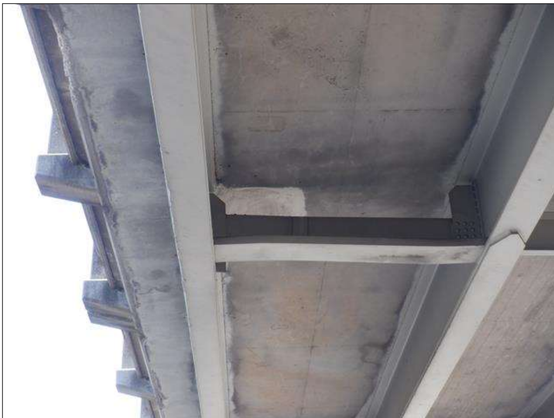
Span 2 Beam 1: PREVIOUS IMPACT DAMAGE AT FIRST INTERMEDIATE DIAPHRAGM WITH SCRAPES IN COVER PLATE, 12 INCHES COLUMN CHANNEL ADDED AT DIAPHRAGM.
