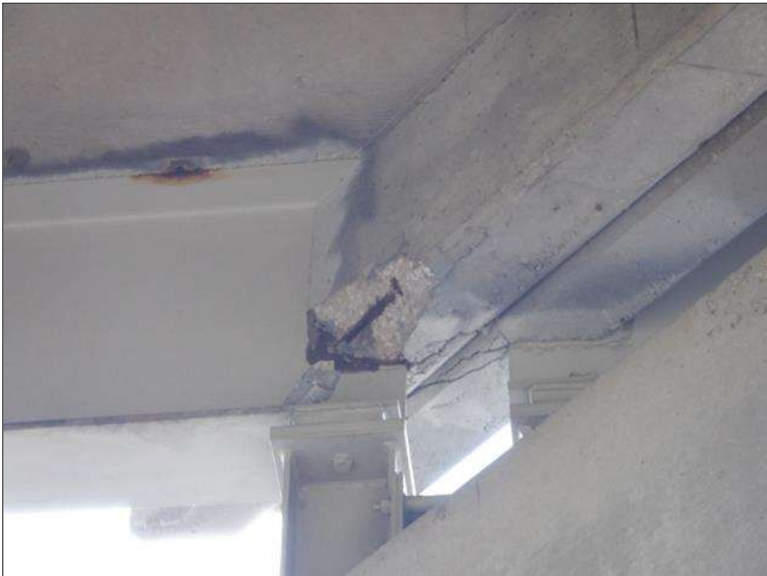
Span 4 Deck: PAR. BAY 3 DIAPHRAGM ADJACENT TO BEAM 4 SPALL WITH EXPOSED REBAR 1 FOOT X 4 INCHES X 4 INCHES. 5 PERCENT SECTION LOSS.
