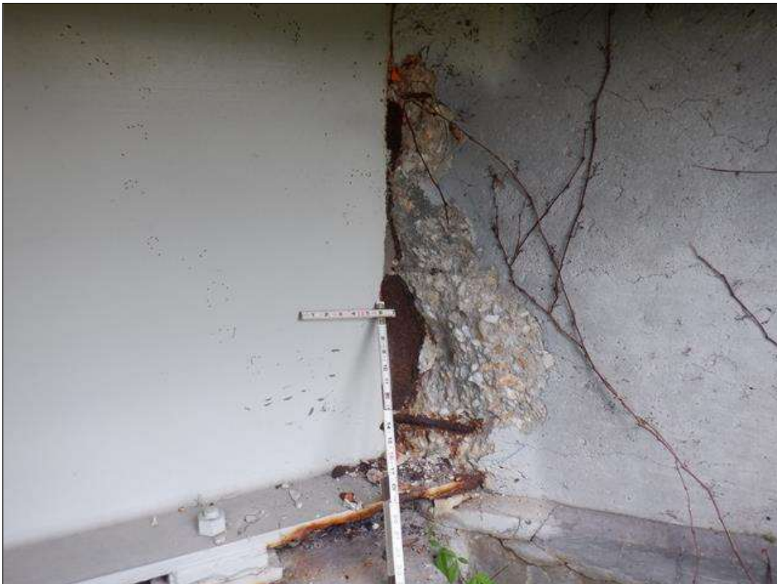
End Bent 1 Abutment: 20 INCHES HIGH X 12 INCHES WIDE X 3 INCHES DEEP SPALL WITH EXPOSED REBAR IN BACKWALL ADJACENT TO THE LEFT SIDE WEB OF BEAM 1, NO SECTION LOSS.
