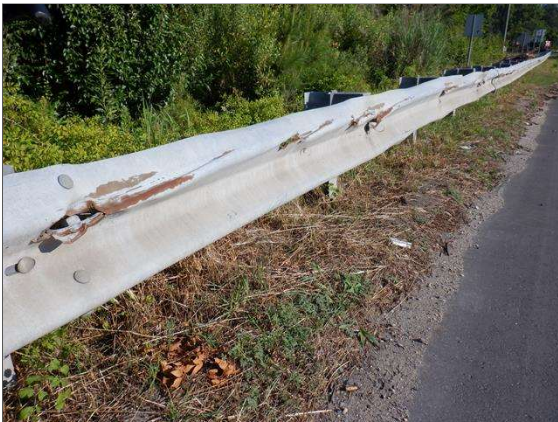
PAR. AT NORTHWEST APPROACH GUARDRAIL 2 AREAS OF UP TO 45 FEET OF IMPACT DAMAGE WITH LOSS OF CONNECTION AT 4 POSTS AND DISTORTION UP TO 3 INCHES.
