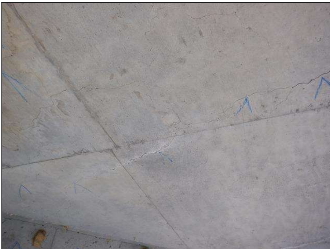
Span 4 Deck: 5 FEET OF 1/16 INCH TRANSVERSE AND MAP-CRACKING IN BOTTOM OF DECK BAY 3
