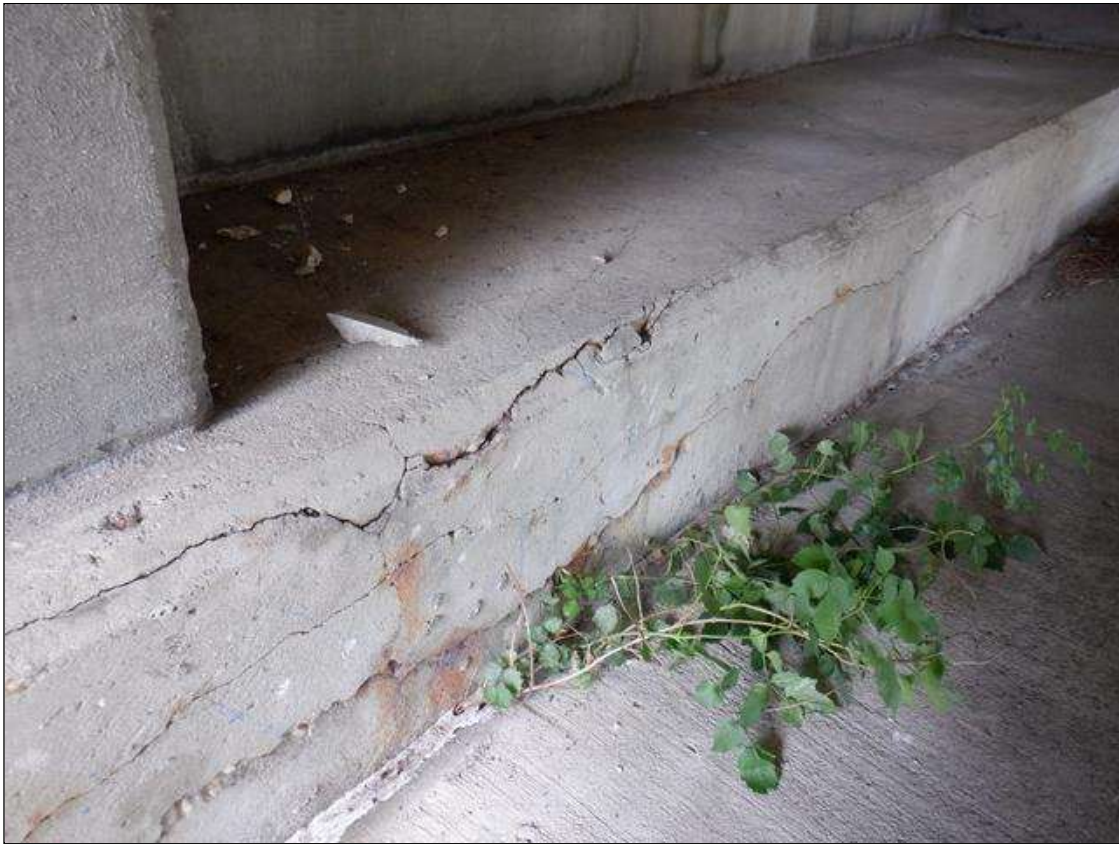
End Bent 2 Cap 1: 8 FEET LONGITUDINAL UP TO 1/8 INCH CRACKING FACE AND TOP WITH 6 FEET X 6 INCHES DELAMINATION AND RUST STAINING IN BAY 1.
