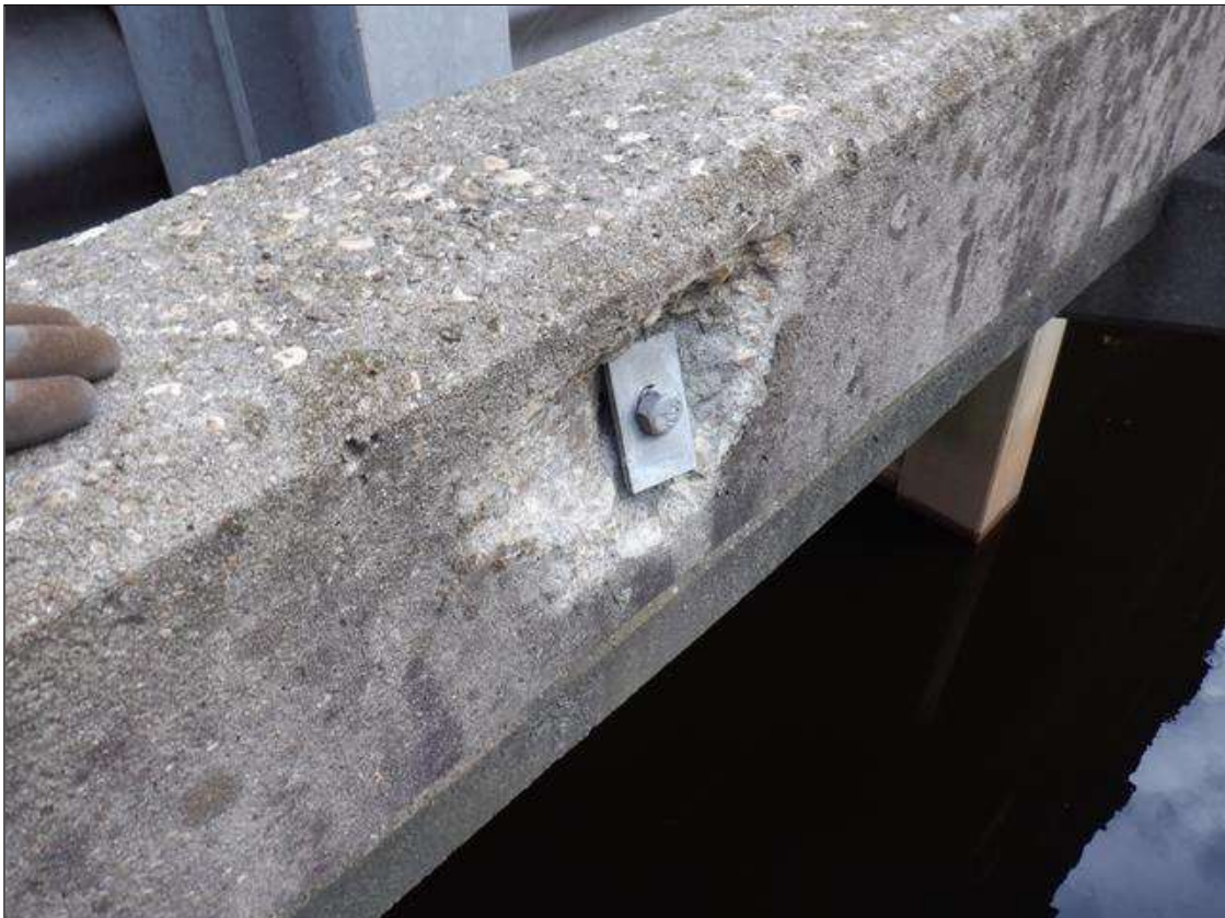
Span 2 Right Concrete Rail: 9 INCHES X UP TO 9 INCHES X 1 INCHES SPALL IN OUTSIDE FACE AT MIDSPAN.
