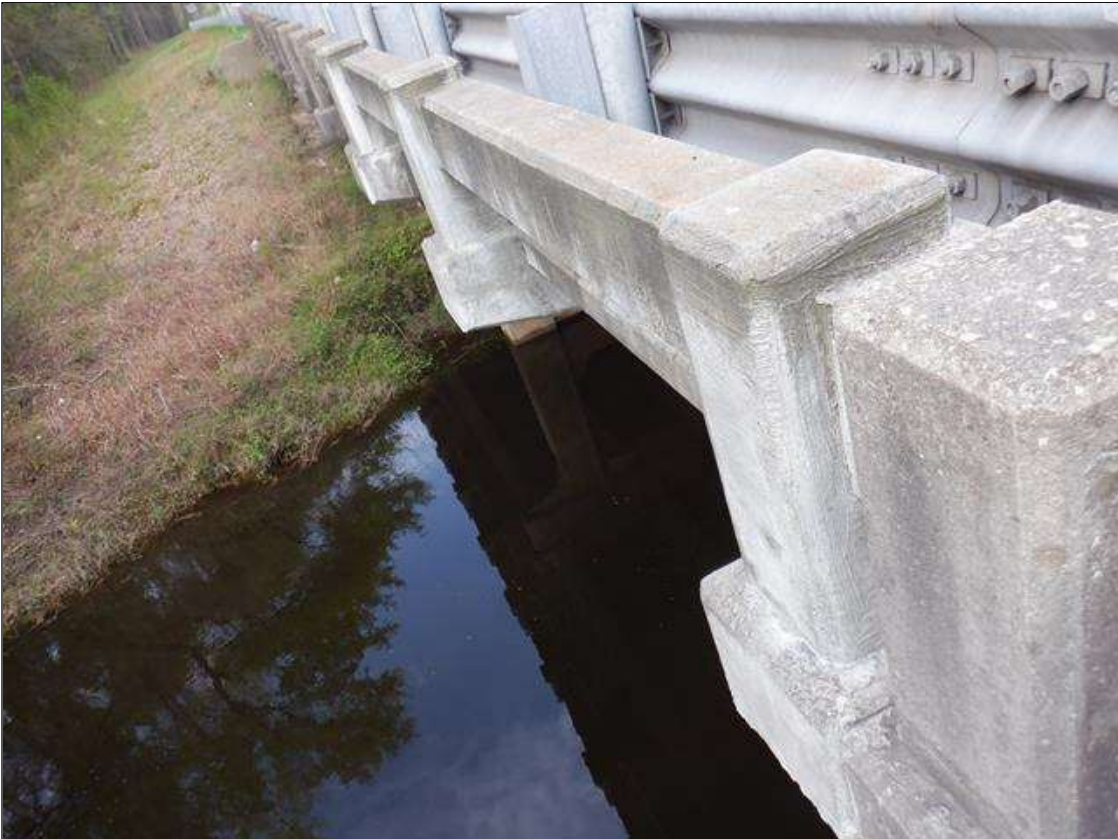
Span 2 Right Concrete Rail: 16 FEET OF REPAIRED SECTION OF CONCRETE RAIL AT BENT 2.
