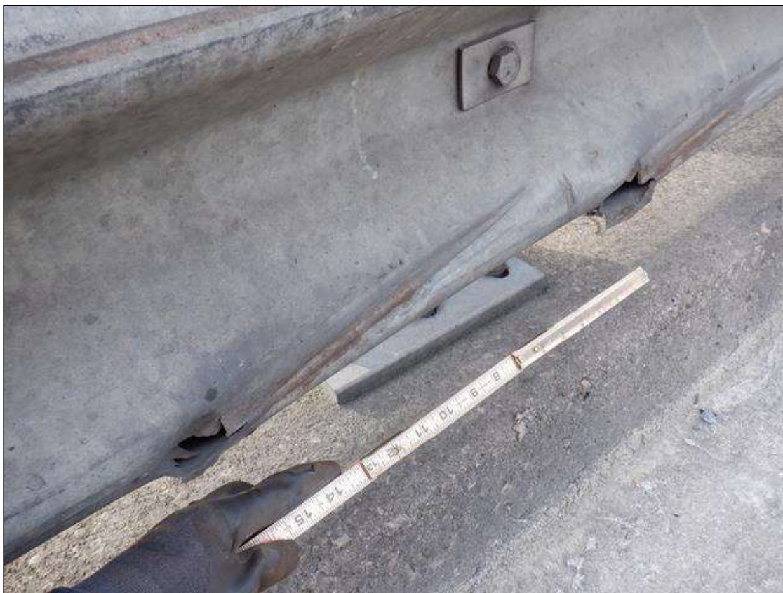
Span 3 Right Metal Rail: (PAR) 50 FEET OF IMPACT DAMAGE WITH 8- UP TO 4 INCHES X 1.5 INCHES GOUGES.
