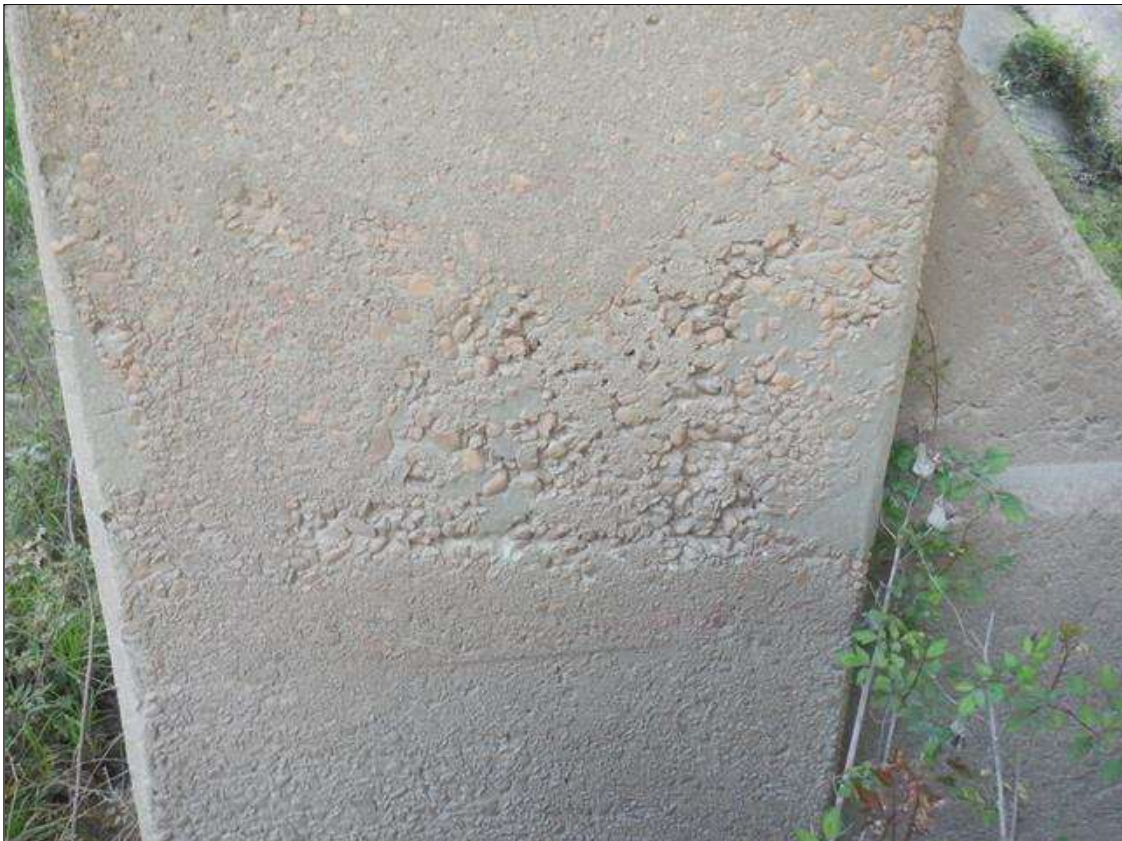
Bent 3 Pile 1: 15 INCHES X UP TO 19 INCHES AREA OF UP TO 1/2 INCHES HONEYCOMBING IN NORTH AND SOUTH FACES, AT STRUT HEIGHT.
