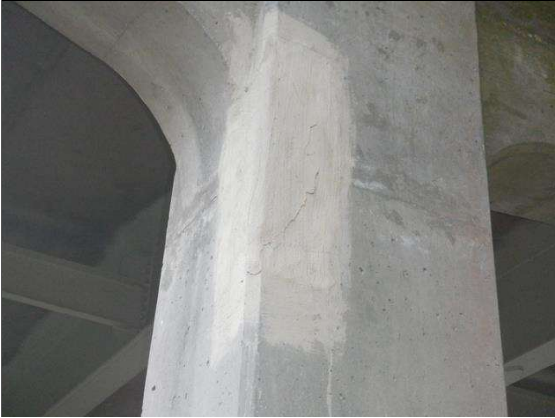
Bent 3 Pile 1: 24 INCHES X UP TO 7 INCHES X 4 INCHES CRACKED AND DELAMINATED PATCHED AREA WITH UP TO 1/16 INCHES CRACKING IN SOUTH FACE, 2 FEET FROM BOTTOM OF CAP.
