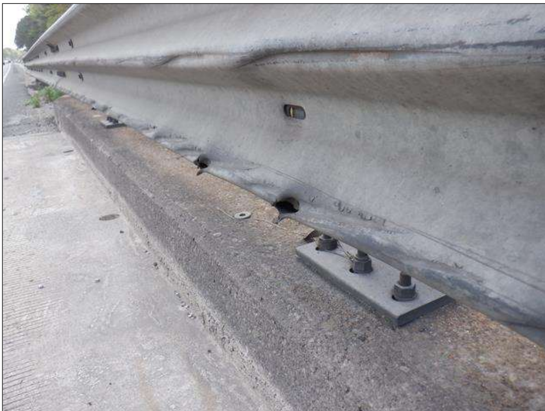
Span 4 Right Metal Rail: (PAR) 51 FEET OF IMPACT DAMAGE WITH 5- UP TO 3 INCHES X 1 INCHES GOUGES.
