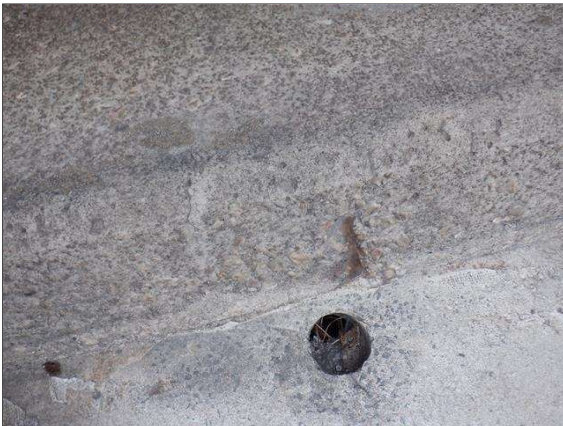
Span 4 Left Concrete Rail: 2 INCHES X 6 INCHES X UP TO 1/2 INCHES SPALL WITH EXPOSED REINFORCING IN EAST FACE OF CURB, NEAR MIDSPAN.
