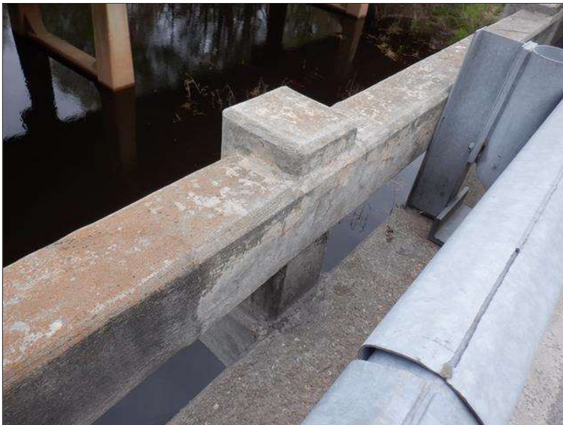
Span 2 Left Concrete Rail: 10 FEET X 1 FEET X 1 FEET CRACKED PATCHED AREA WITH UP TO 1/64 INCHES CRACKING AT MIDSPAN.
