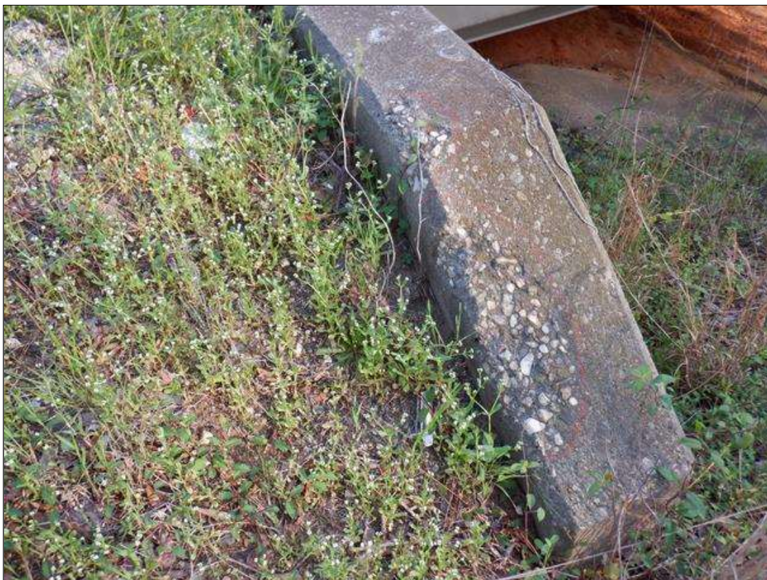
WINGWALL: 2- UP TO 18 INCHES X 5 INCHES X 3 INCHES SPALLS IN TOP OF SOUTHEAST WINGWALL.
