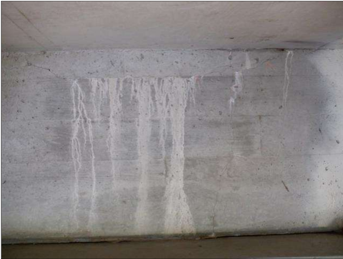
End Bent 2 Abutment: 24 SQUARE FEET OF UP TO 1/8 INCHES HORIZONTAL AND VERTICAL CRACKS, SOME WITH EFFLORESCENCE, IN ALL BAYS. (PHOTO TAKEN IN BAY 2)
