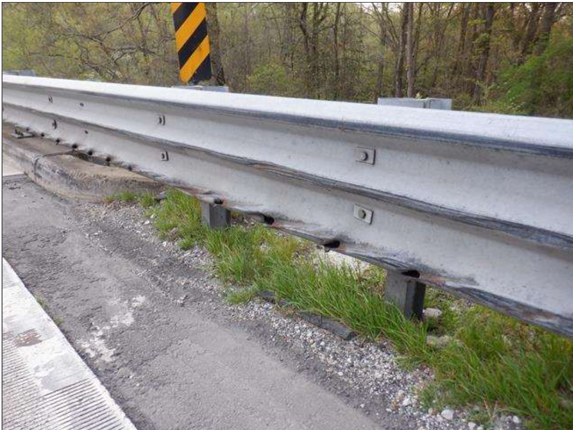
General Comments and Misc. Items: (PAR) 15 FEET OF IMPACT DAMAGE WITH 11- UP TO 4 INCHES X 2 INCHES GOUGES IN SOUTHEAST GUARDRAIL AT END BENT 1.
