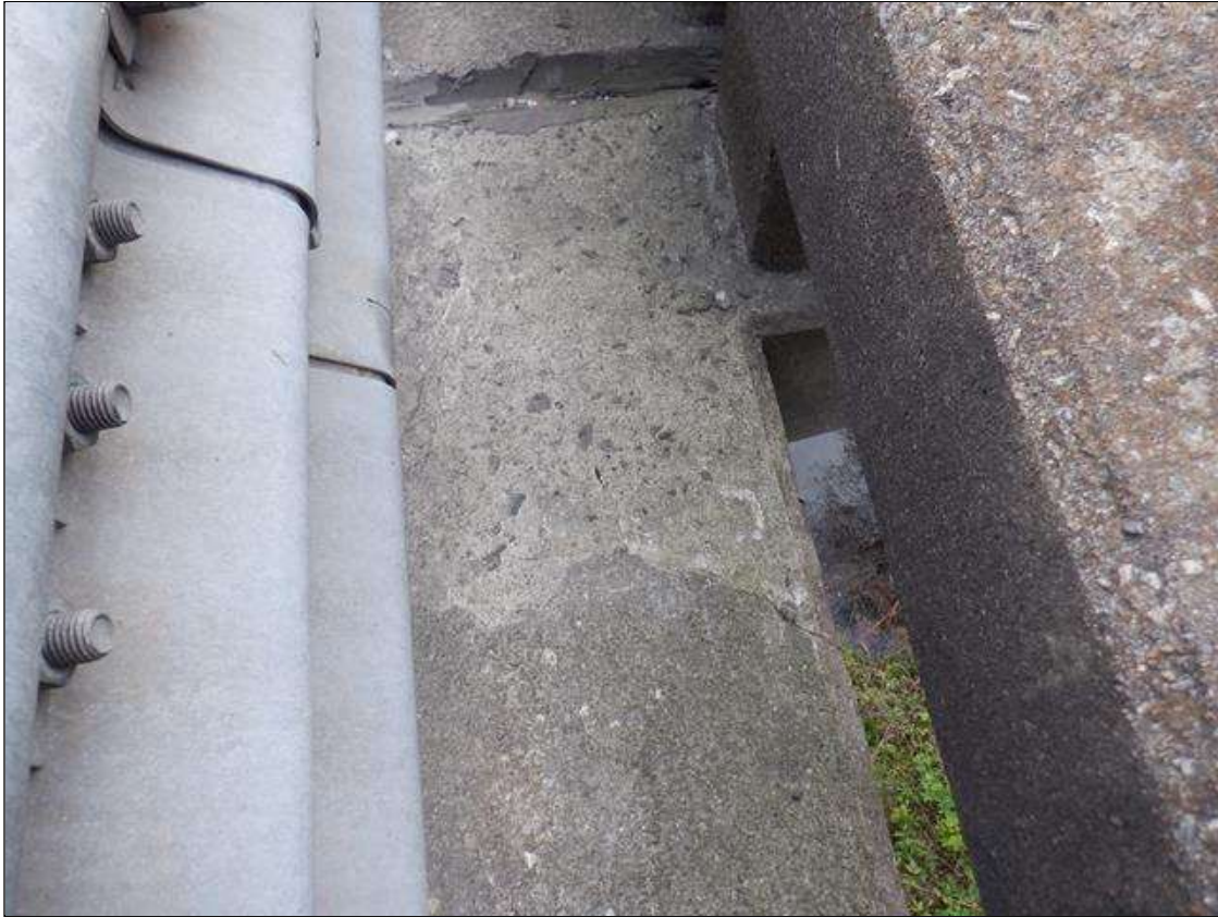
Span 1 Right Concrete Rail: 2 FEET X UP TO 2 FEET CRACKED PATCHED AREA WITH UP TO 1/32 INCHES CRACKING IN CURB AT BENT 1.
