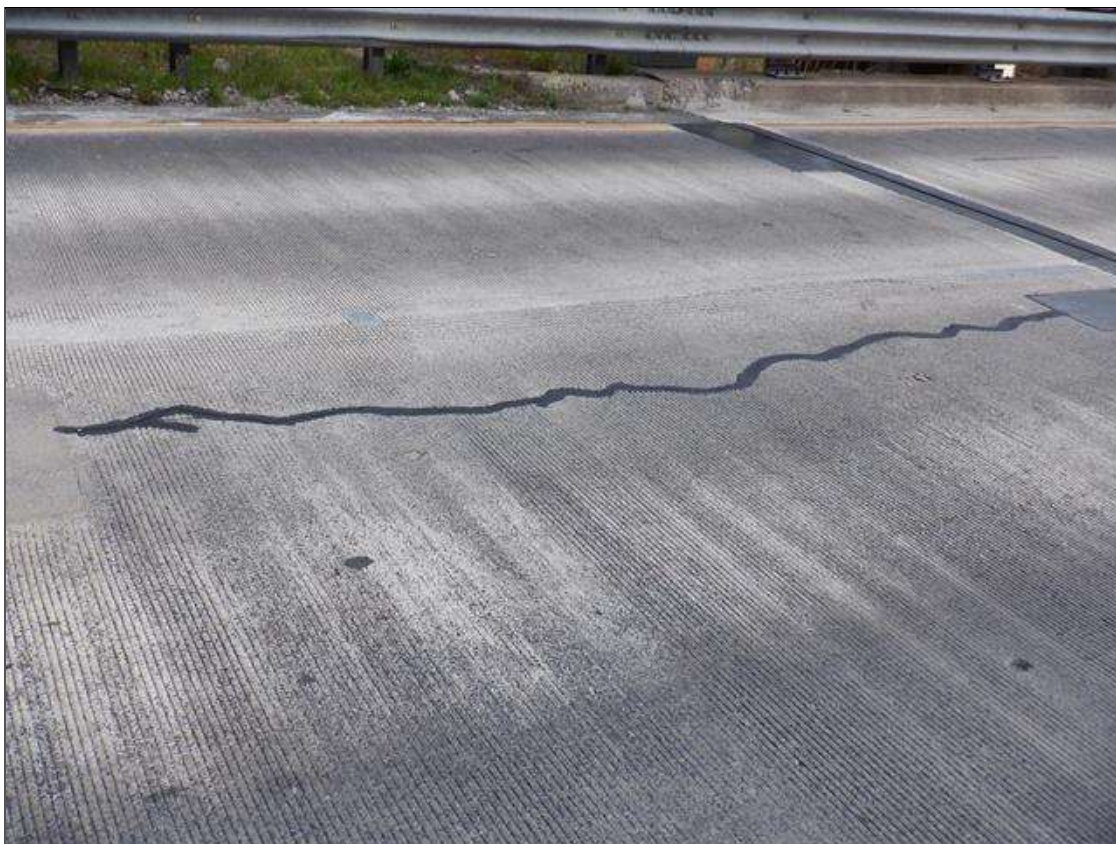
Approach 1 : 15 FEET SEALED LONGITUDINAL CRACK NEAR CENTERLINE
