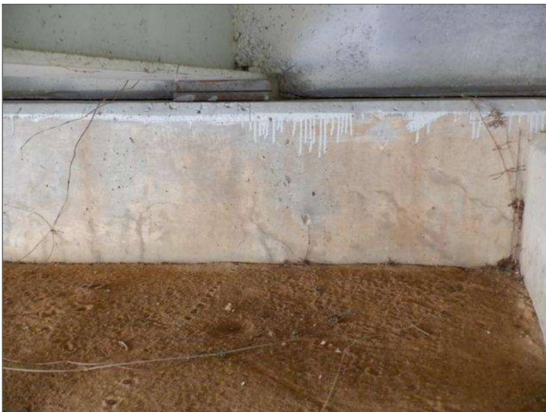
End Bent 2 Cap 1: 12 FEET X UP TO 2 FEET AREA OF UP TO 1/32 INCHES MAP CRACKING, BEGINNING AT WEST END.
