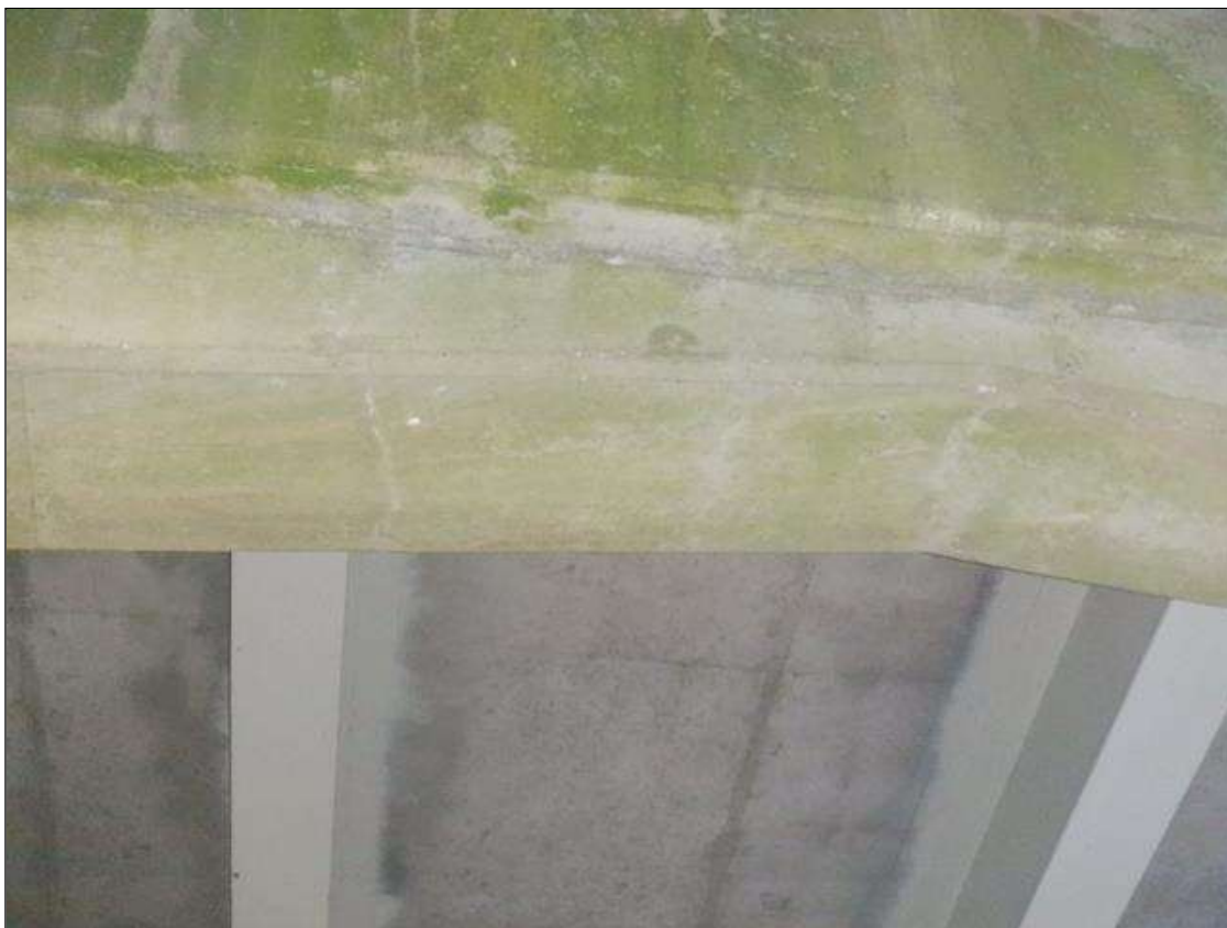
Bent 2 Cap 1: (3) UP TO 20 INCHES X 1/64 INCHES TRANSVERSE CRACKS, SOME WITH EFFLORESCENCE, ON BOTTOM OF CORBEL BETWEEN COLUMNS 1 AND 2.
