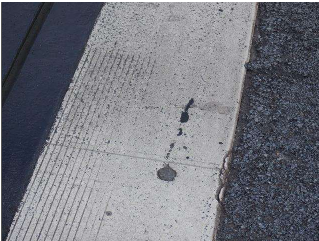
Approach 2 : 18 INCHES X UP TO 1/64 INCHES LONGITUDINAL CRACK IN EAST LANE
