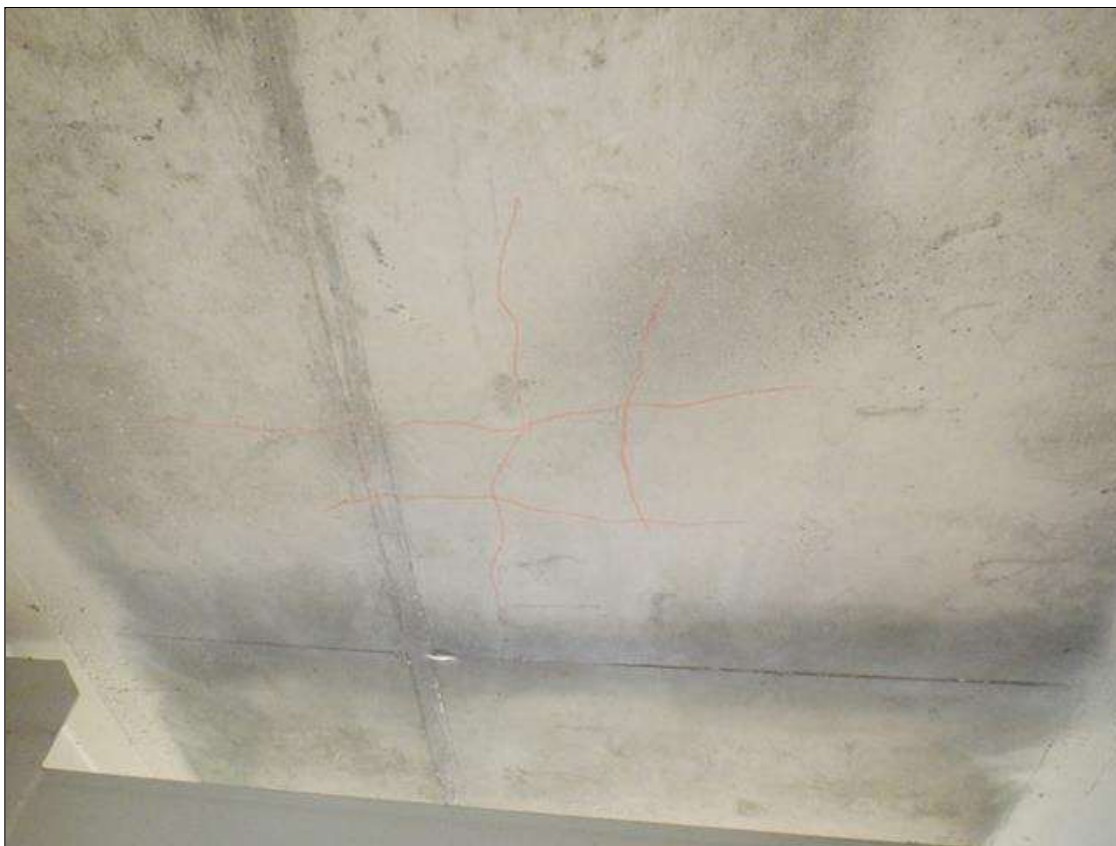
Span 1 Deck: 750 SQUARE FEET OF UP TO 1/32 INCHES MAP CRACKING AT RANDOM THROUGHOUT UNDERSIDE. (PHOTO TAKEN IN BAY 1)
