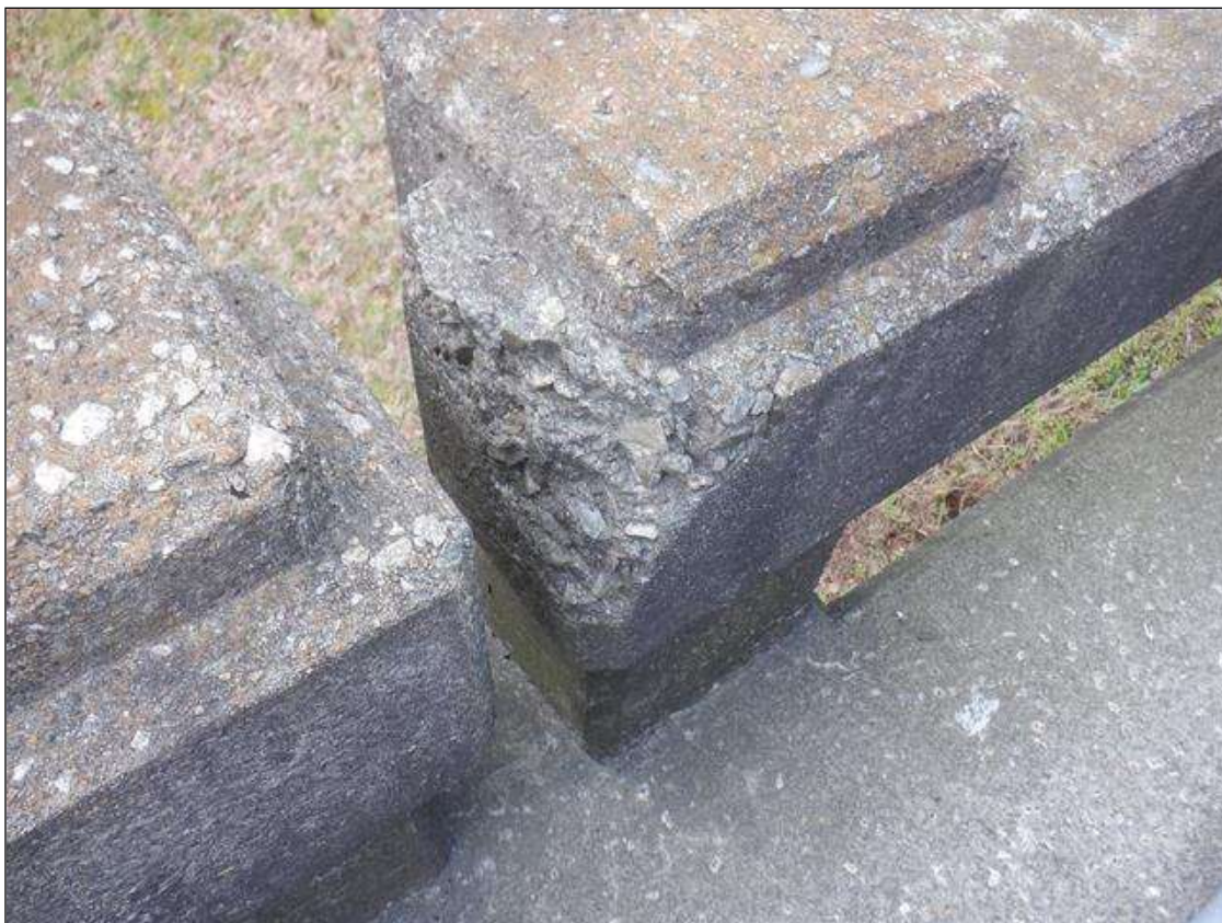
Span 1 Right Concrete Rail: 4 INCHES X 7 INCHES X UP TO 6 INCHES SPALL AT POST 2.
