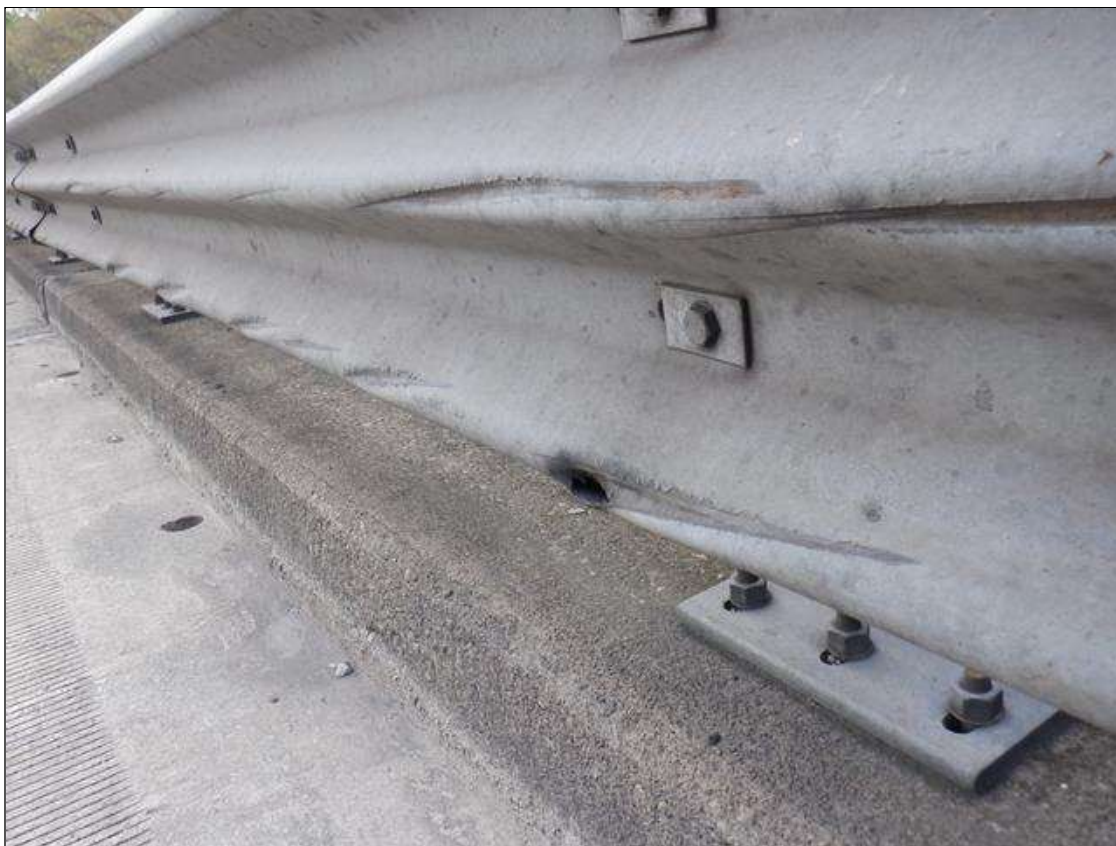
Span 1 Right Metal Rail: (PAR) 52 FEET OF IMPACT DAMAGE WITH SCRAPES AND 4- UP TO 3 INCHES X 1.5 INCHES GOUGES.
