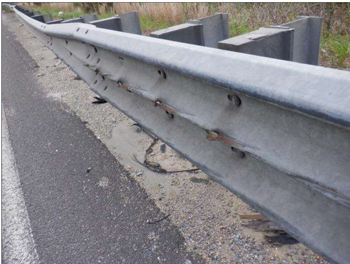
General Comments and Misc. Items: (PAR) 15 FEET OF IMPACT DAMAGE WITH 4- UP TO 3 INCHES X 1 INCHES GOUGES IN NORTHEAST GUARDRAIL, 50 FEET FROM END BENT 2.
