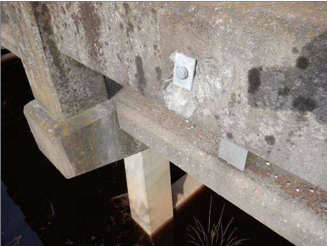
Span 4 Right Concrete Rail: 5- UP TO 7 INCHES X 6 INCHES X 1 INCHES SPALLS IN OUTSIDE FACE OF RAIL. (PHOTO TAKEN NEAR MIDSPAN)
