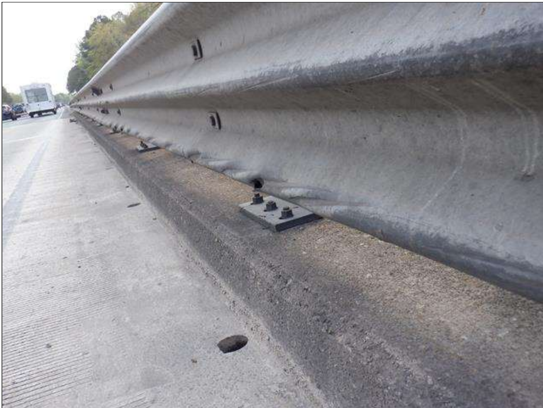
Span 3 Right Metal Rail: (PAR) 50 FEET OF IMPACT DAMAGE WITH 8- UP TO 4 INCHES X 1.5 INCHES GOUGES.
