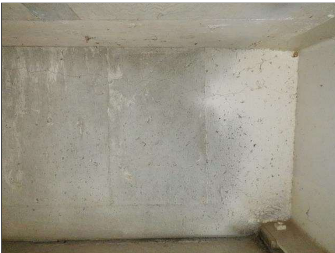
End Bent 1 Abutment: 32 FEET OF UP TO 1/32 INCHES HORIZONTAL AND VERTICAL CRACKS, SOME WITH EFFLORESCENCE. (PHOTO TAKEN IN BAY 2)
