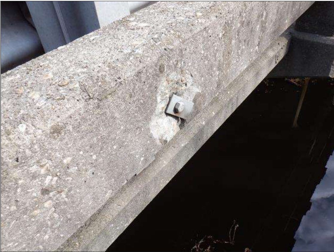
Span 3 Right Concrete Rail: (3) UP TO 9 INCHES X 9 INCHES X 1 INCHES SPALLS IN OUTSIDE FACE. (PHOTO TAKEN NEAR BENT 2)
