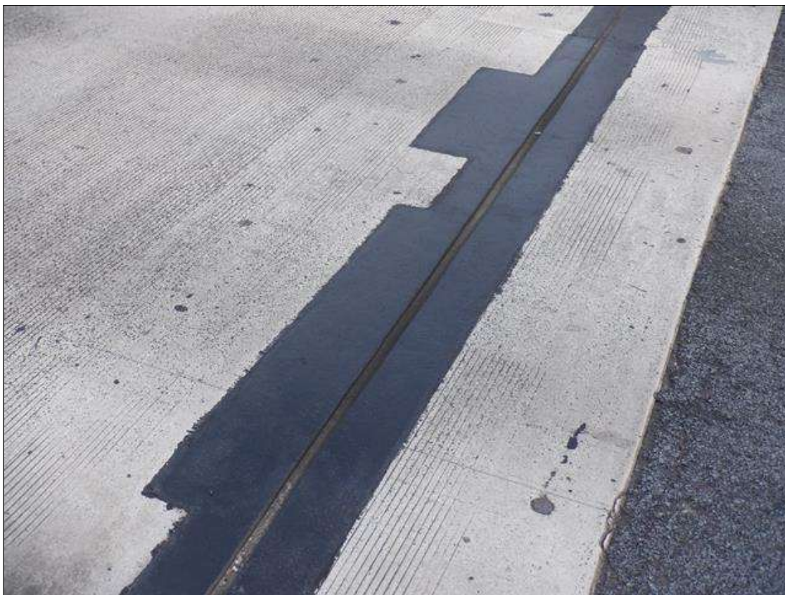
Span 4 Expansion Joint at End Bent 2: 2- UP TO 7 FEET X 18 INCHES PATCHED AREAS ALONG SOUTH EDGE IN EAST LANE.
