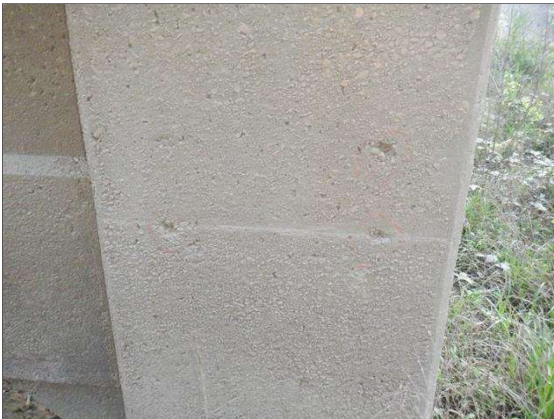
Bent 3 Pile 2: (3) UP TO 2 INCHES X 2 INCHES X 1/2 INCHES SPALLS IN SOUTH FACE, 11 FEET FROM BOTTOM OF CAP.
