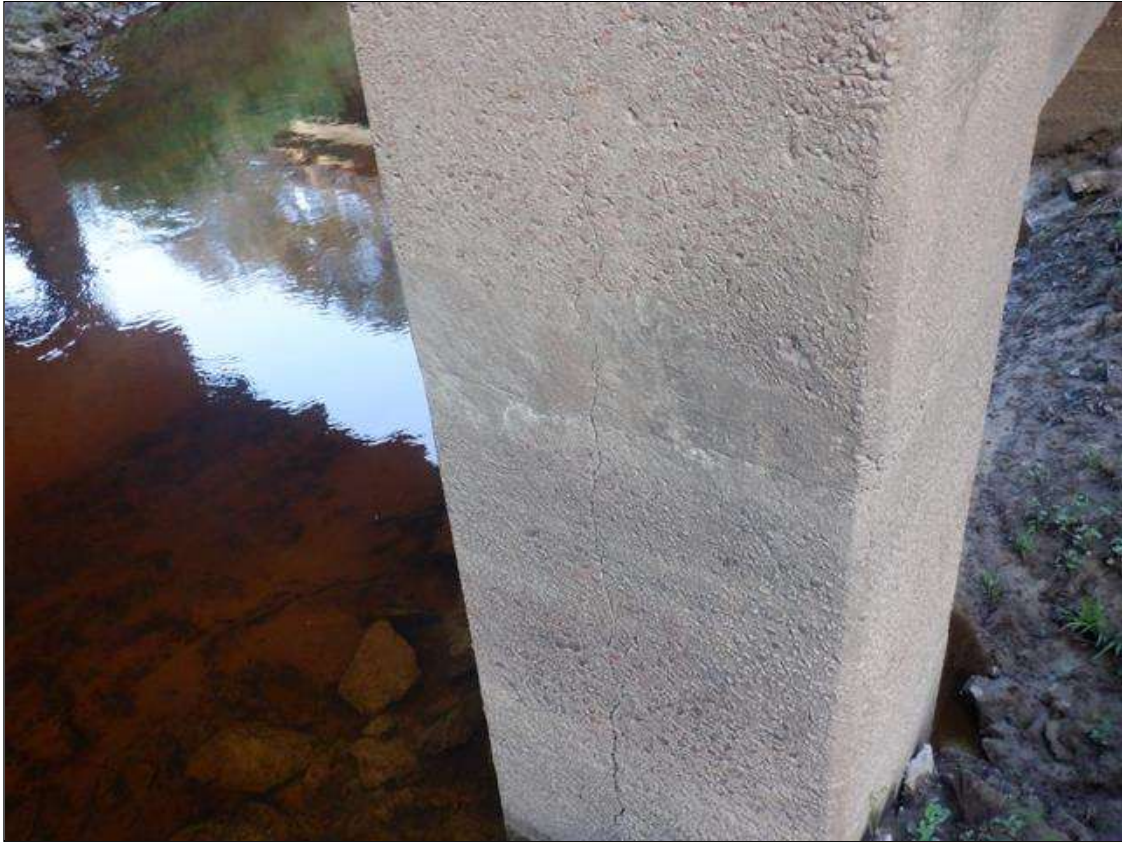
Bent 2 Pile 2: 2- UP TO 6 FEET X 1/8 INCHES VERTICAL CRACKS ON NORTH AND EAST FACE, 13 FEET FROM BOTTOM OF CAP.
