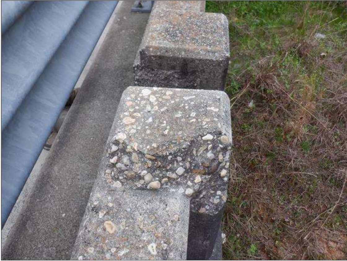
Span 1 Left Concrete Rail: 2- UP TO 4 INCHES X 10 INCHES X 7 INCHES SPALLS WITH EXPOSED REINFORCING IN TOP OF POSTS, 17 FEET FROM END BENT 1.
