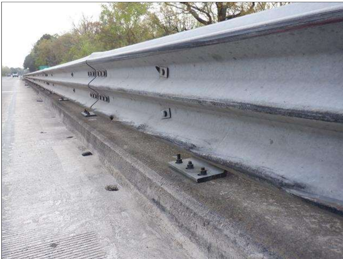
Span 1 Right Metal Rail: (PAR) 52 FEET OF IMPACT DAMAGE WITH SCRAPES AND 4- UP TO 3 INCHES X 1.5 INCHES GOUGES.
