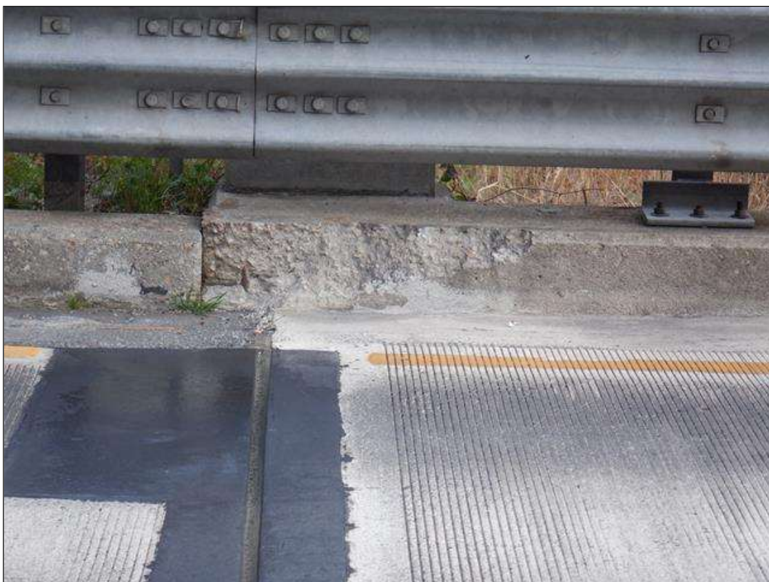
Span 1 Left Concrete Rail: 35 INCHES X UP TO 9 INCHES X 2 INCHES SPALL WITH EXPOSED REBAR IN CURB AT END BENT 1.
