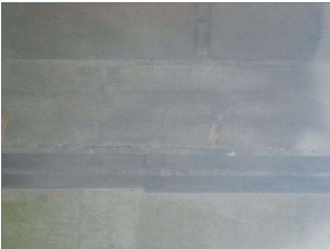
Span 4 Deck: 5- FULL HEIGHT X UP TO 1/32 INCHES VERTICAL CRACKS IN BENT 3 BAY 1 DIAPHRAGM. (BAYS 2 AND 3 SIMILAR)
