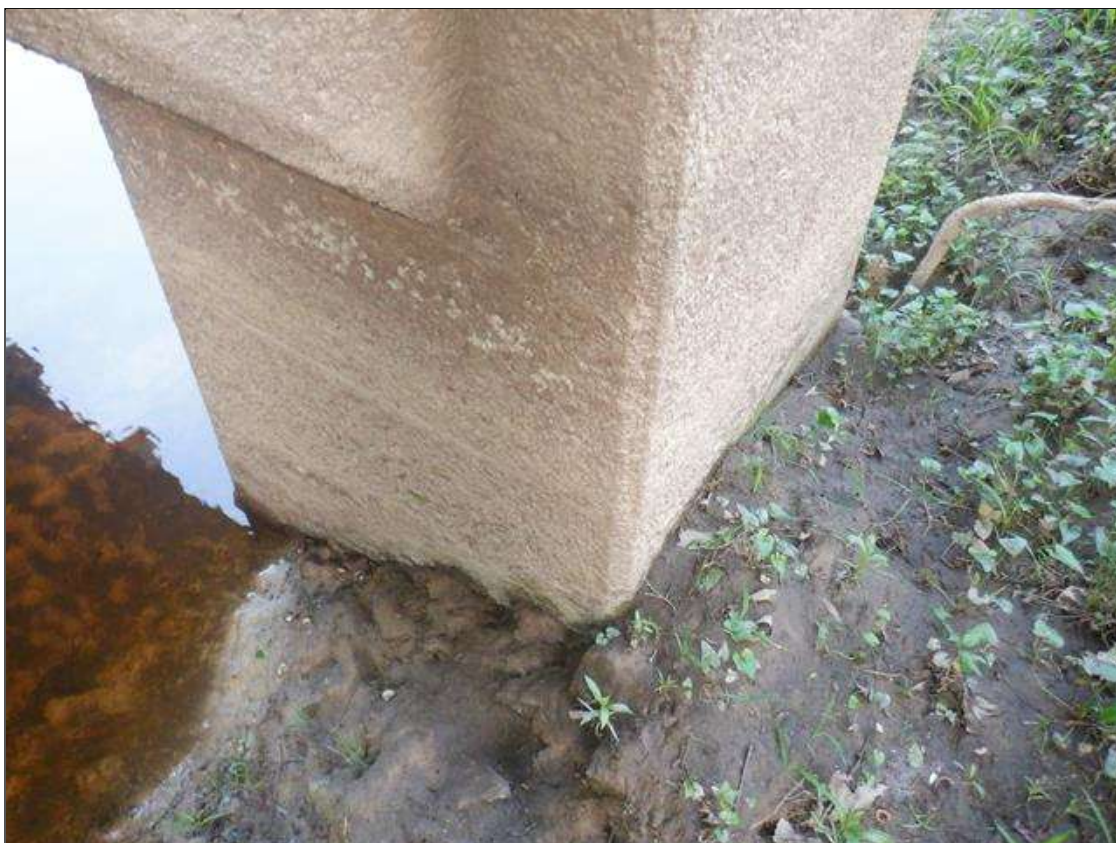
Bent 2 Pile 1: 4 FEET ABRASION/WEAR WITH EXPOSED COARSE AGGREGATE, 12 FEET FROM BOTTOM OF CAP.
