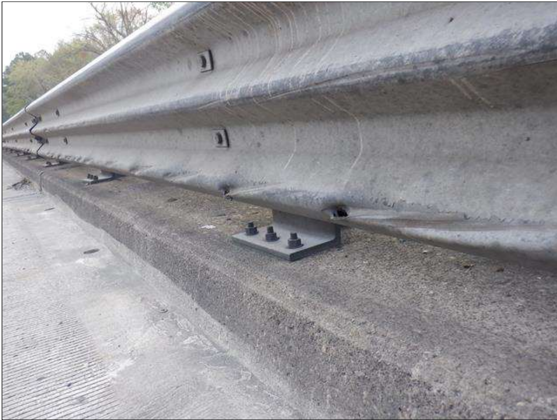
Span 2 Right Metal Rail: (PAR) 50 FEET OF IMPACT DAMAGE WITH SCRAPES AND 4- UP TO 2 INCHES X 1 INCHES GOUGES.
