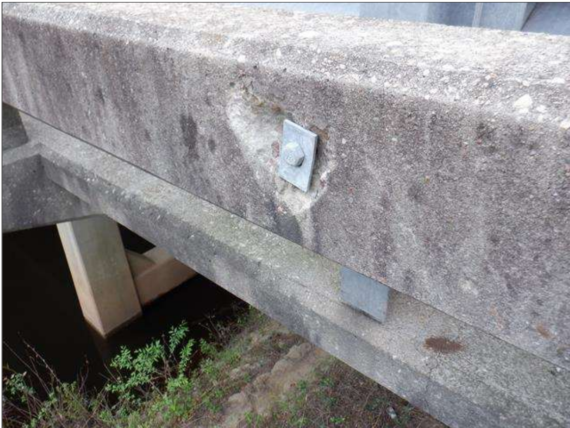
Span 1 Left Concrete Rail: (5) UP TO 7 INCHES X 9 INCHES X 1 INCHES SPALLS ON OUTSIDE FACE AT BOLT LOCATIONS.
