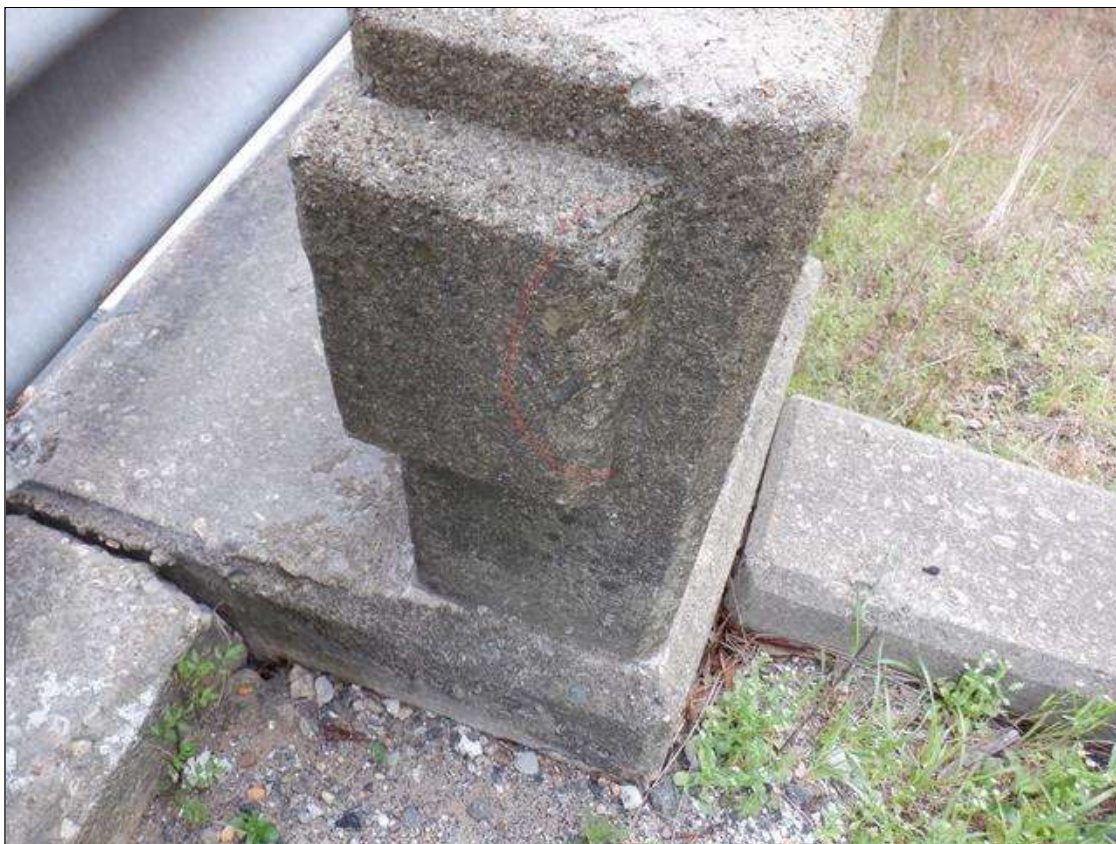
Span 1 Right Concrete Rail: 2 INCHES X UP TO 3 INCHES X 1/2 INCHES SPALL ON END POST AT END BENT 1.
