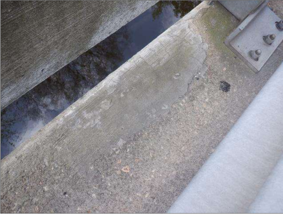
Span 2 Right Concrete Rail: 36 INCHES X UP TO 9 INCHES CRACKED PATCHED AREA WITH UP TO 1/64 INCHES CRACKING IN CURB NEAR BENT 2.
