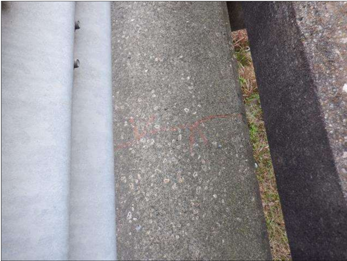
Span 1 Right Concrete Rail: (6) UP TO 1/64 INCHES TRANSVERSE AND WRAPAROUND CRACKS AT RANDOM THROUGHOUT CURB AND RAIL.
