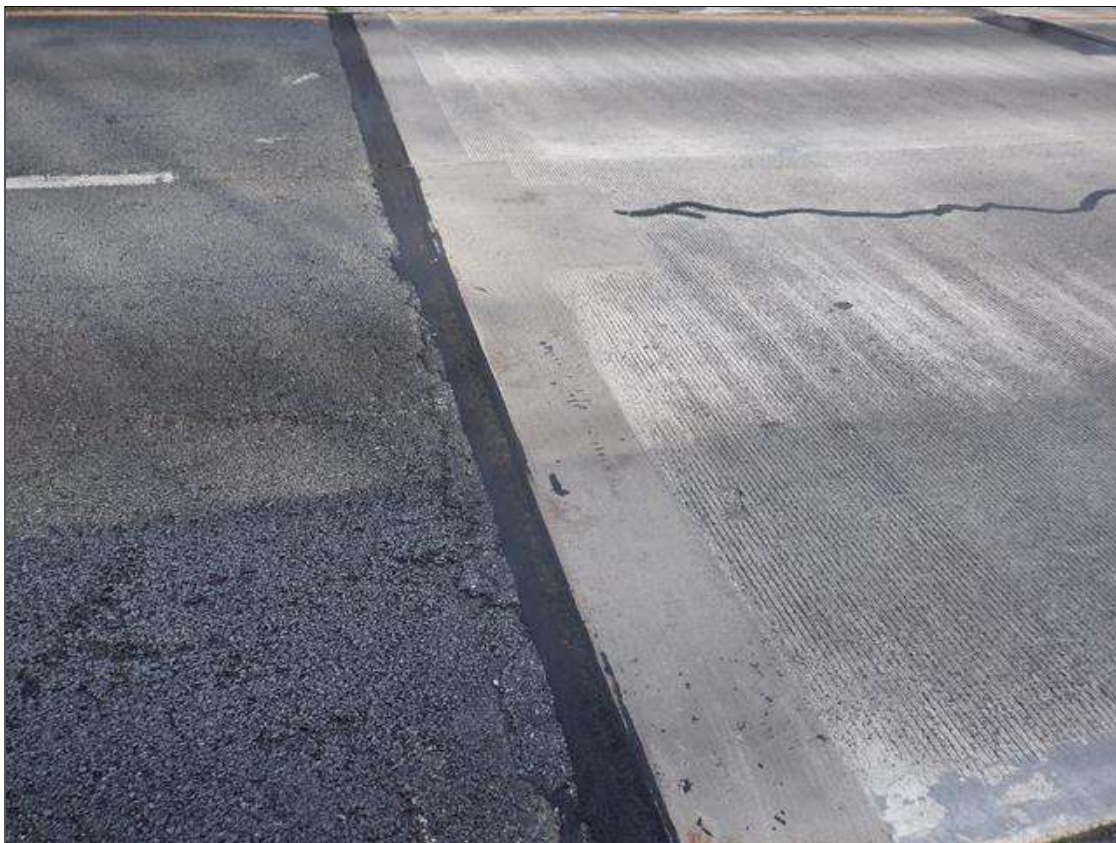
Approach 1 : FULL WIDTH X UP TO 3 FEET PATCHED AREA IN SOUTH END.
