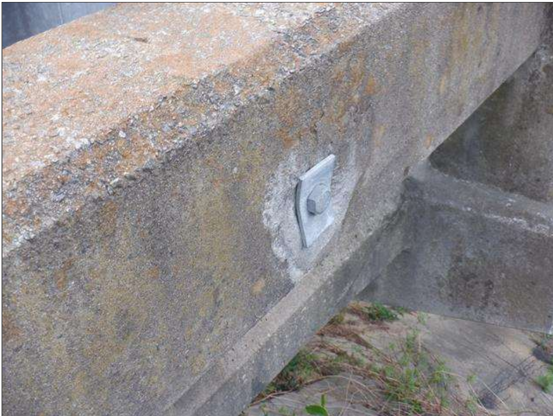
Span 4 Left Concrete Rail: (2) UP TO 8 INCHES X 8 INCHES X 1 INCHES SPALLS IN OUTSIDE FACE OF RAIL. (PHOTO TAKEN NEAR END BENT 2)
