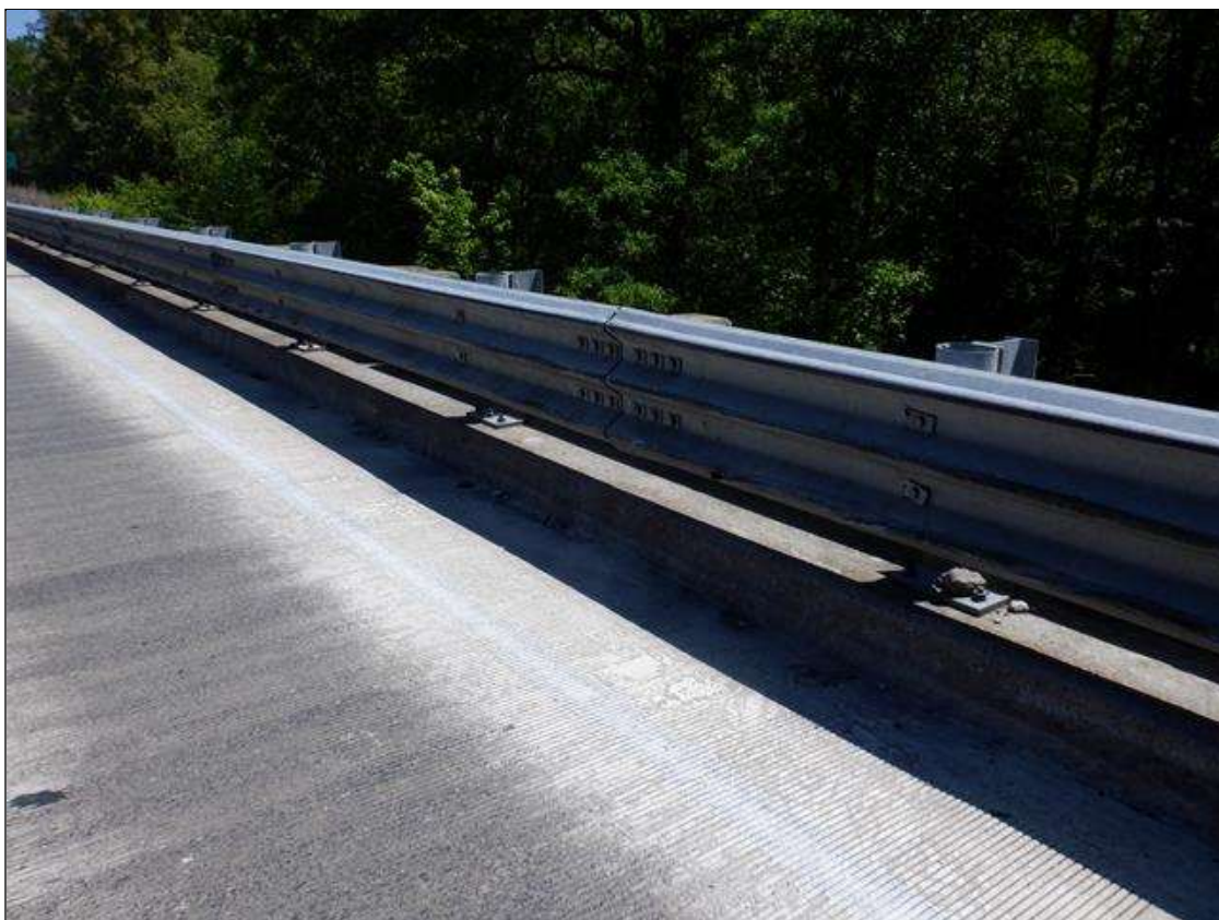
Span 1 Right Bridge Rail: (PAR) 52' OF DAMAGE TO METAL BRIDGE RAIL.
