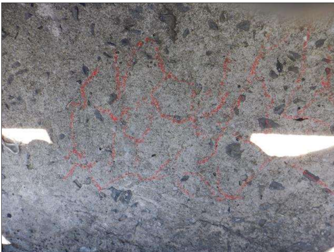
Span 1 Right Bridge Rail: 2' x 2' cracked patched area on concrete curb at Bent 1
