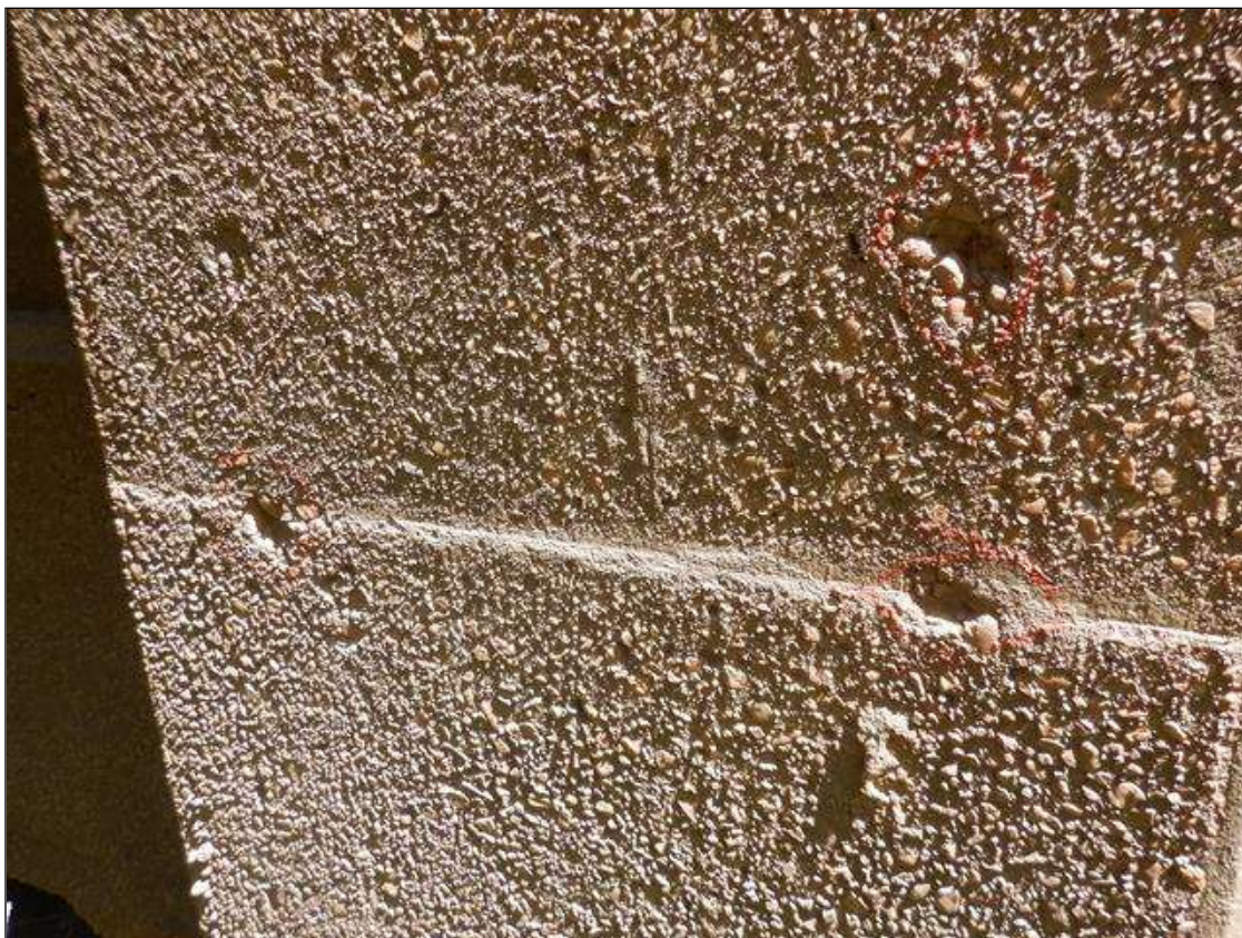
Bent 3 Pile 2: (3) up to 2" x 2" x 1/2" deep spalls on Span 3 face, 11' from bottom of cap
