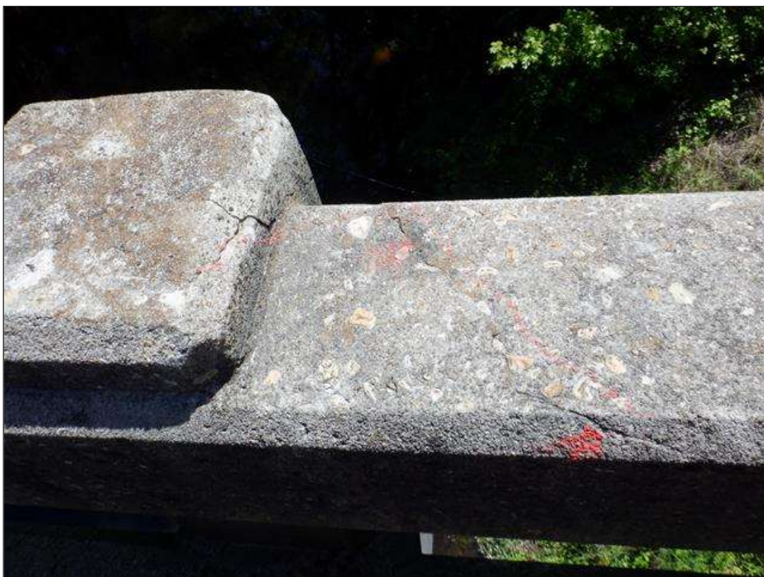
Span 2 Right Bridge Rail: 3" x 1/64" longitudinal crack on top of concrete Post 2
