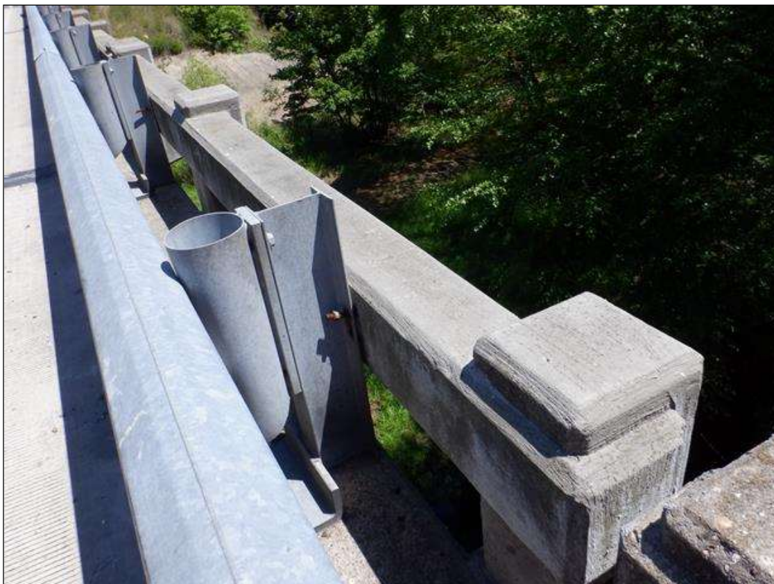
Span 2 Right Bridge Rail: 16' repaired section of concrete rail at Bent 2
