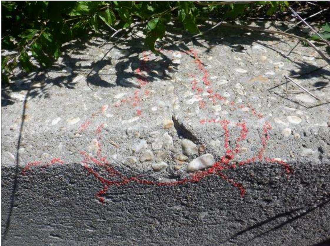
Wingwalls: 5" x 3" x 1" deep spall on Northwest wingwall.
