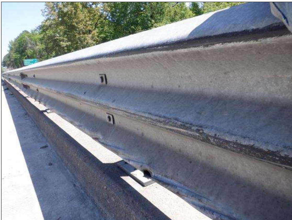
Span 3 Right Bridge Rail: (PAR) 50' OF DAMAGE TO METAL BRIDGE RAIL.
