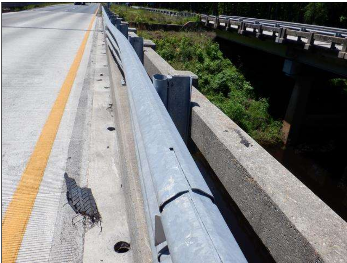
Span 2 Left Bridge Rail: (PAR) 20' impact damage with 2" deflection to the West on metal rail, extending from bent 2.
