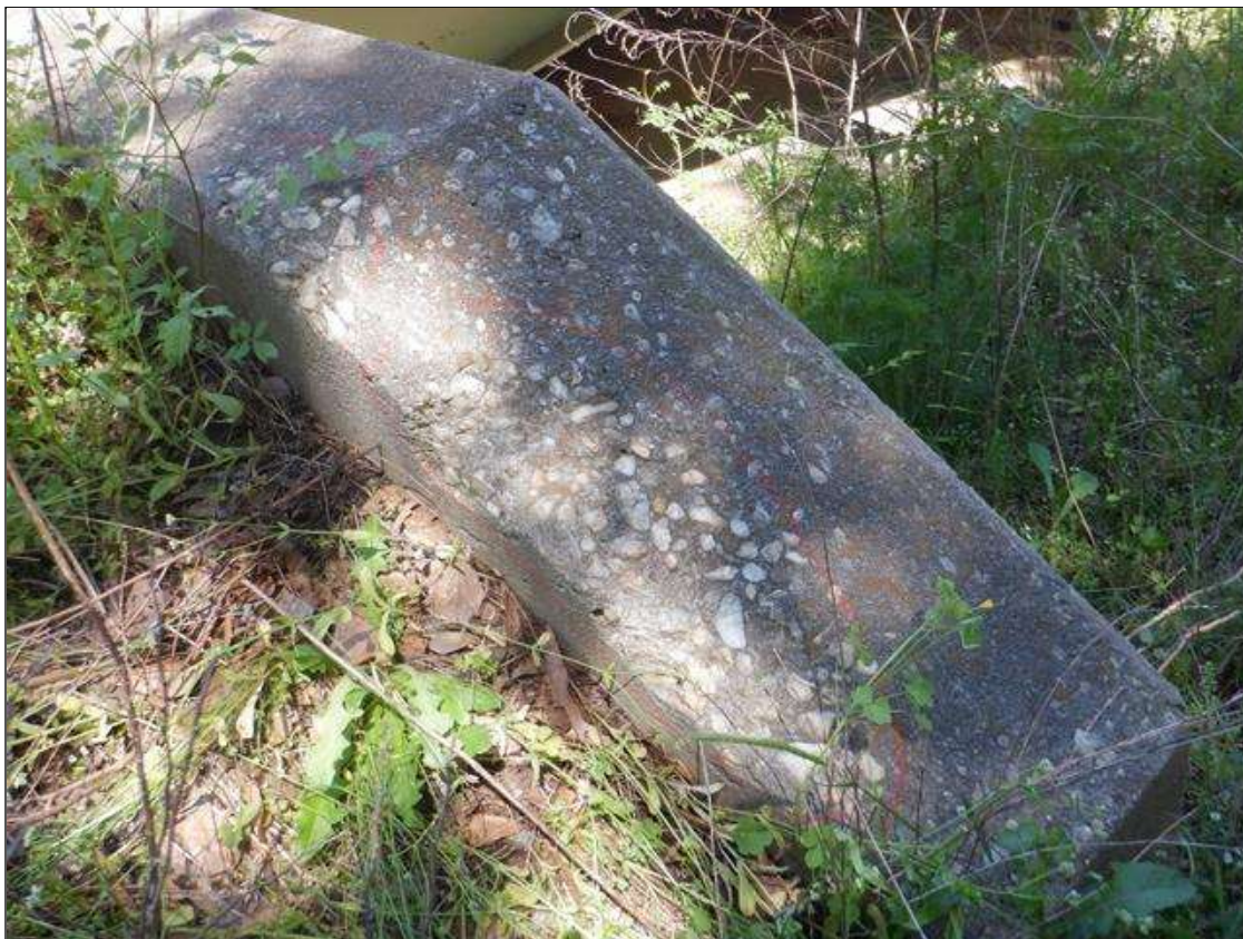
Wingwalls: (2)- up to 18" x 5" x 3" deep spall on top of Southeast wingwall.
