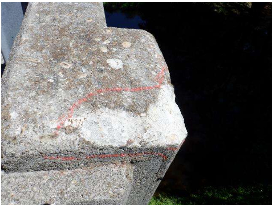
Span 2 Right Bridge Rail: 5" x 6" x 1" deep spall on concrete Post 1
