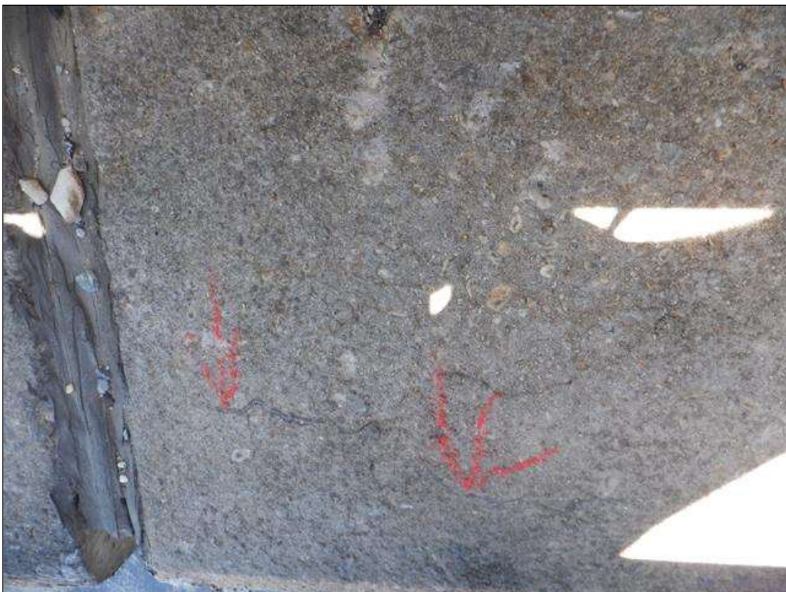
Span 2 Right Bridge Rail: 30" x 1/64" longitudinal cracks on concrete curb at Bent 2
