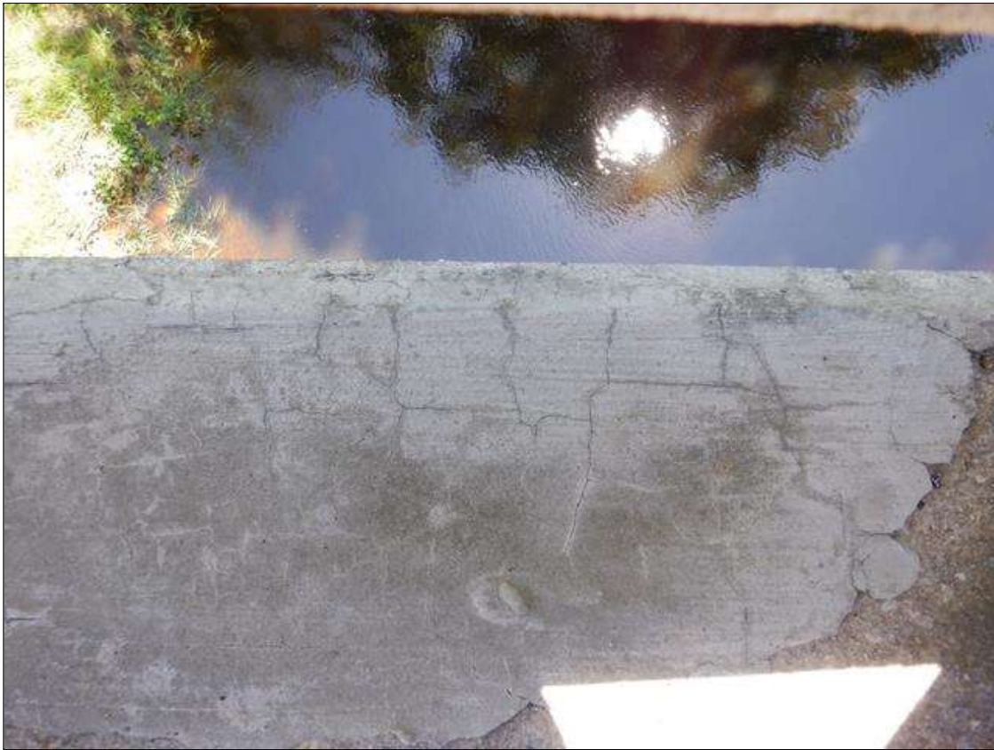
Span 2 Right Bridge Rail: 36" x 9" cracked patched area on concrete curb near Bent 2
