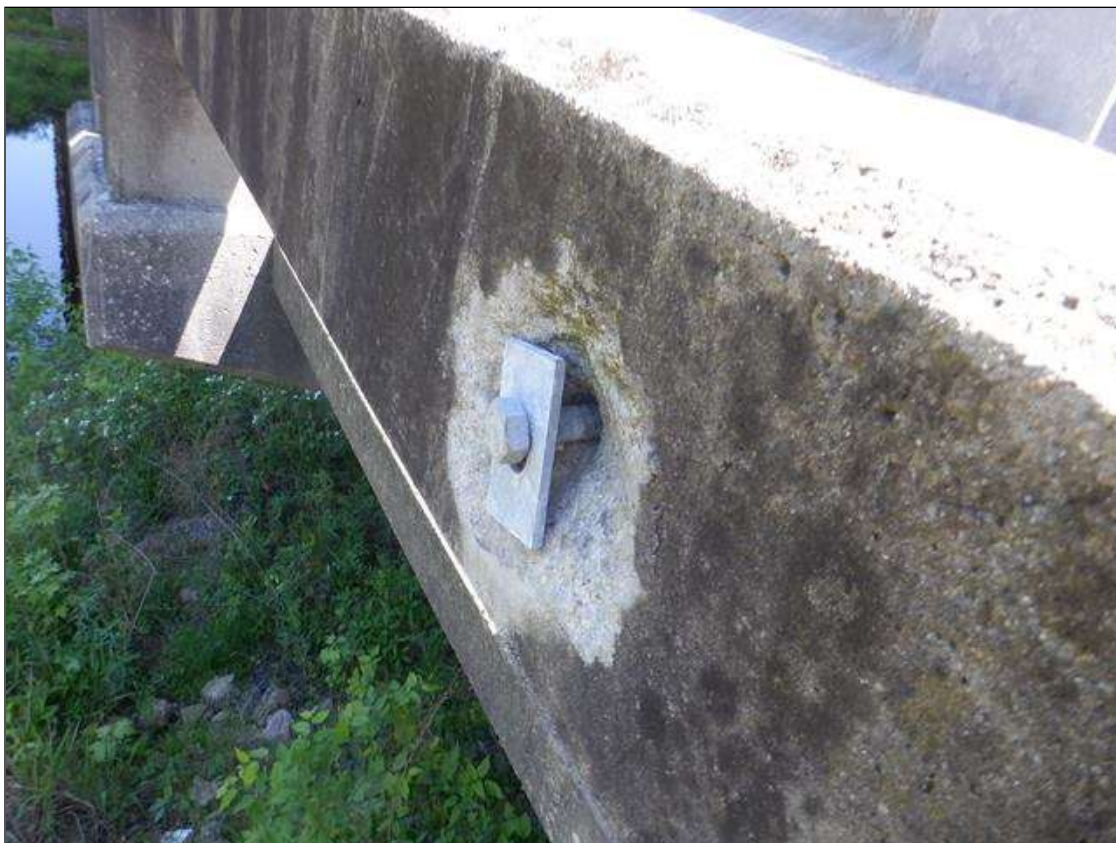
Span 1 Left Bridge Rail: (5) up to 7" x 9" x 1" deep spalls on outside face of concrete rail at bolt locations.
