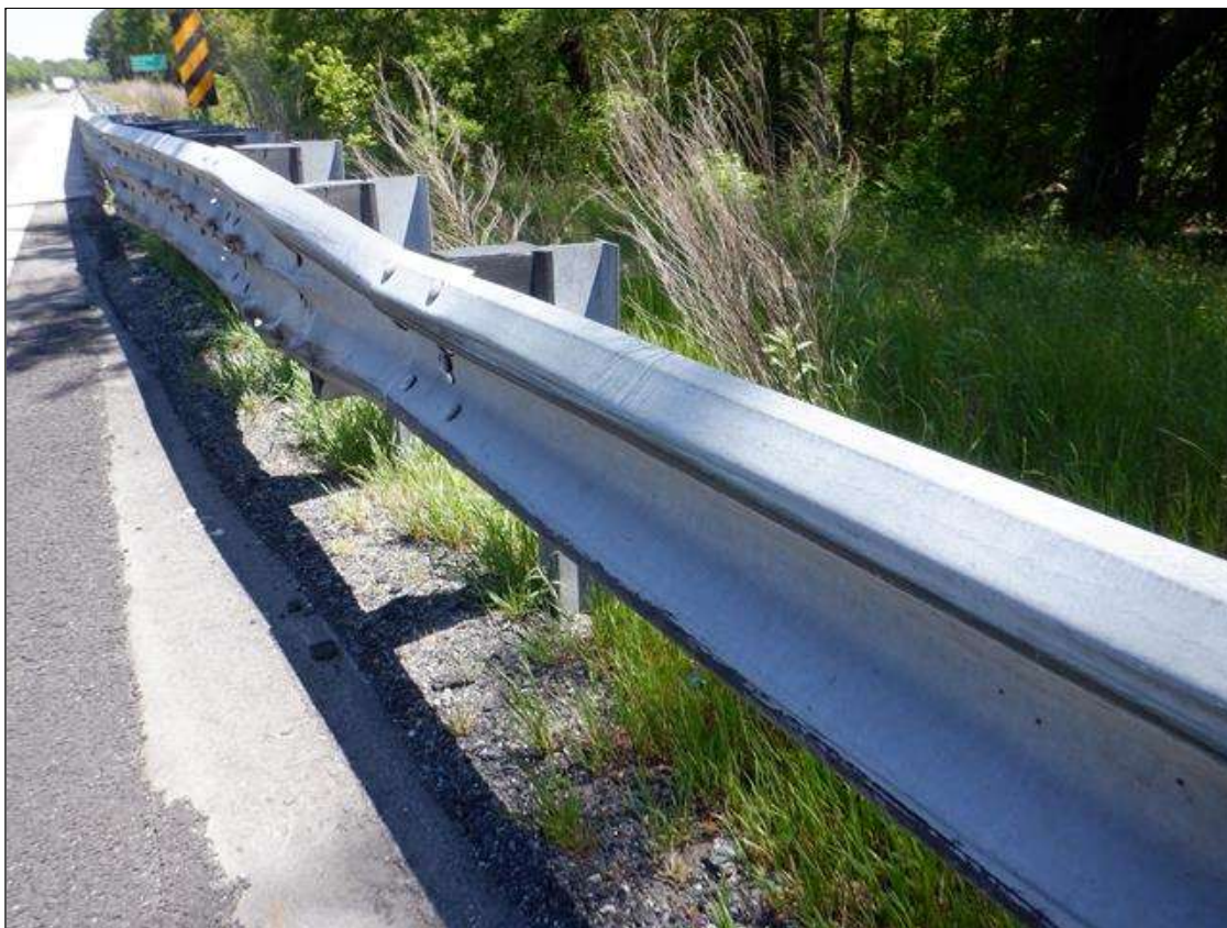
General Comments and Misc. Items: (PAR) 36' OF DAMAGED GUARDRAIL AT SOUTHEAST CORNER, AT END BENT 1.
