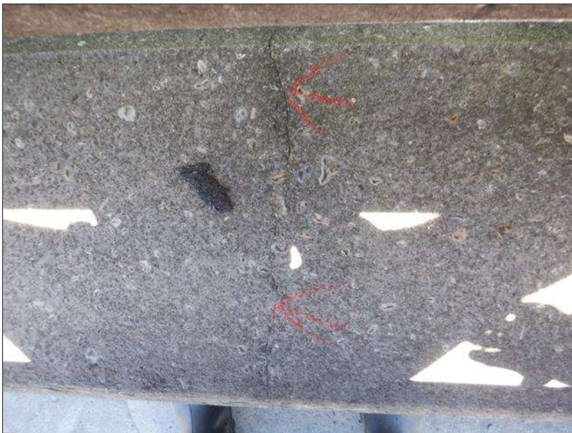
Span 2 Right Bridge Rail: (4) up to 1/64" vertical and transverse cracks on concrete curb and rail
