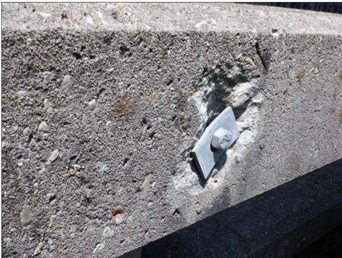
Span 4 Right Bridge Rail: (5) up to 7" x 6" x 1" deep spalls on outside face of concrete rail (PHOTO TAKEN NEAR MIDSPAN)
