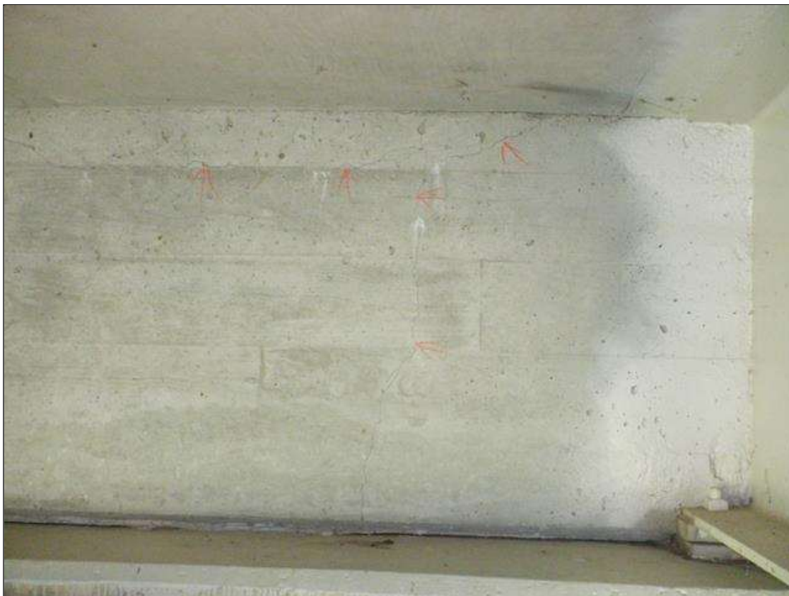
End Bent 2 Abutment/Backwall : HORIZONTAL AND VERTICAL CRACKS UP TO 1/32", SOME WITH EFFLORESCENCE, IN ALL BAYS (PHOTO TAKEN IN BAY 2).
