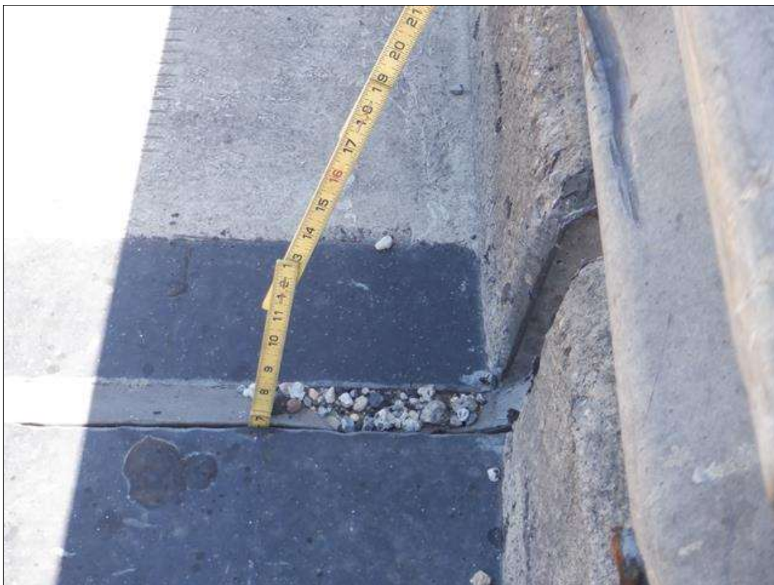
Expansion Joint at Bent 1 : Full length x full depth detached joint material
