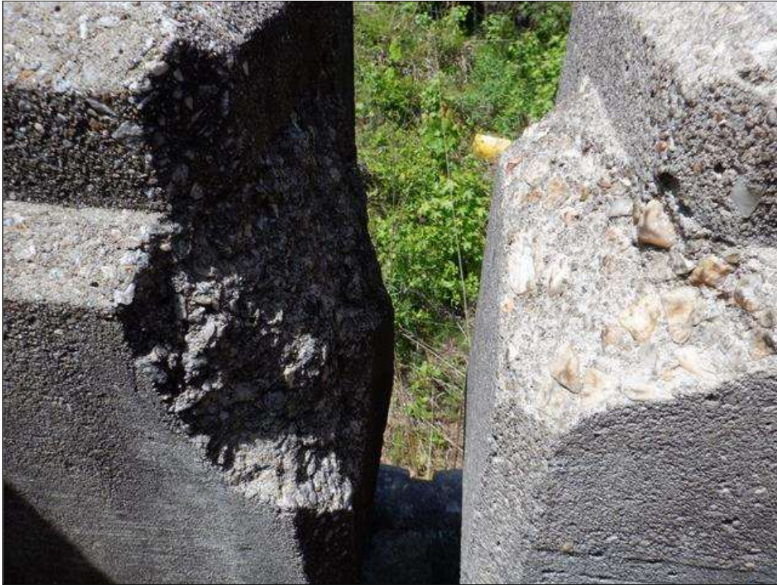
Span 1 Left Bridge Rail: (2)- UP TO 4" X 10" X 7" SPALLS IN TOP OF POSTS, 17' FROM END BENT 1.
