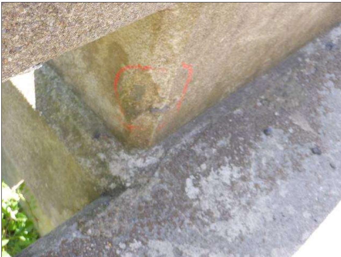
Span 1 Right Bridge Rail: 2" x 3" x 1/2" deep spall on end post at End Bent 1
