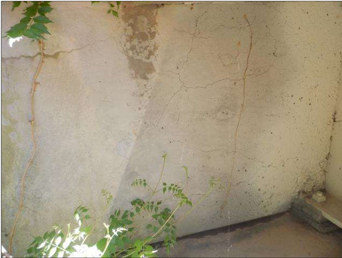
End Bent 1 Abutment/Backwall : 32' OF HORIZONTAL AND VERTICAL CRACKS UP TO 1/32", SOME WITH EFFLORESCENCE (PHOTO TAKEN AT EAST END).
