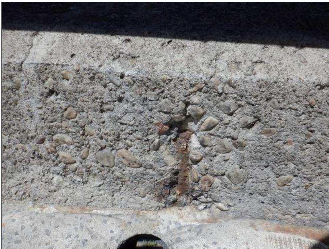
Span 4 Left Bridge Rail: 2" X 6" X 1/2" SPALL WITH EXPOSED REINFORCING, EAST FACE OF CURB, NEAR MIDSPAN.
