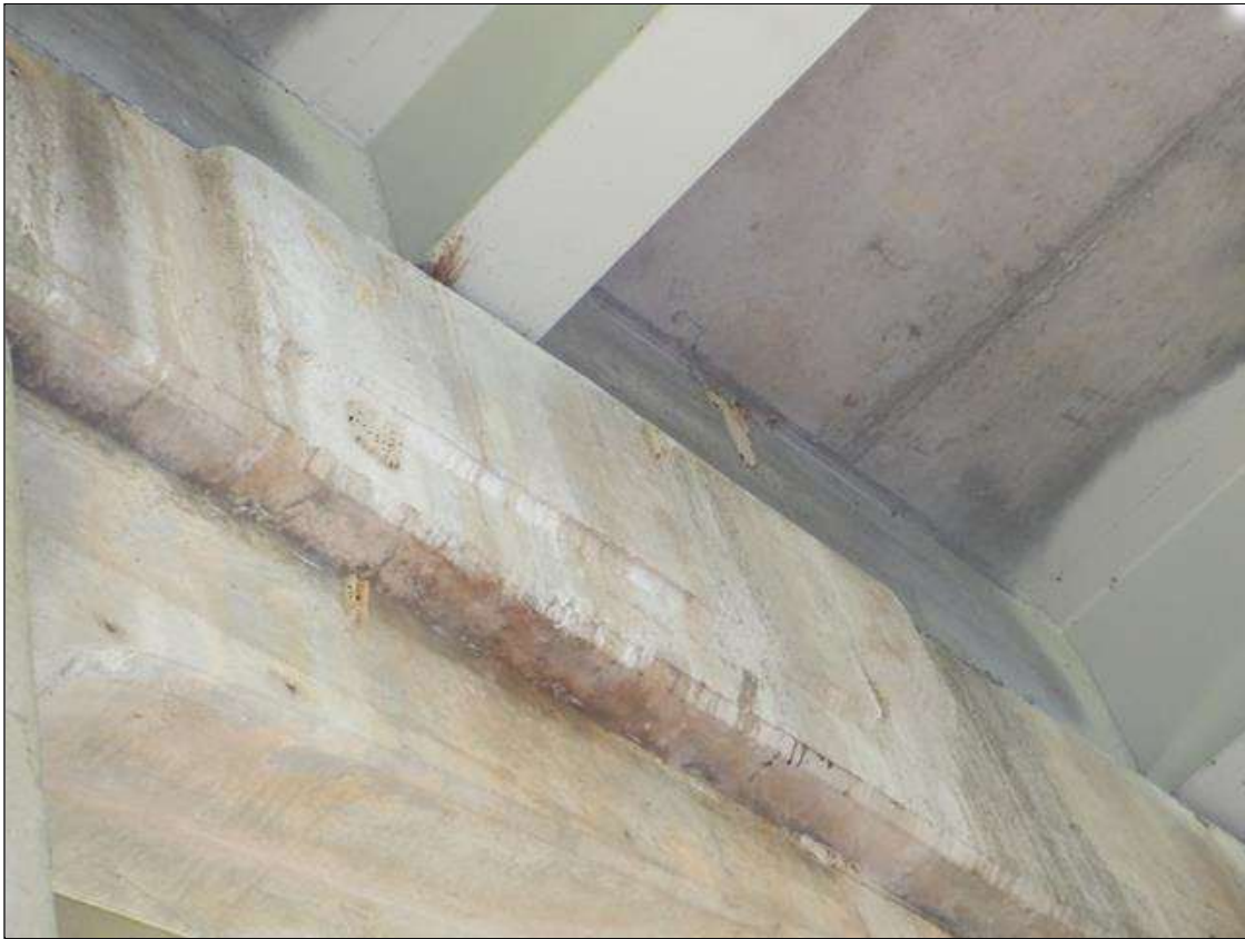
Bent 1 Cap 1: 6' X UP TO 16" PATCHED AREA, NORTH FACE, UNDER BEAM 3.
