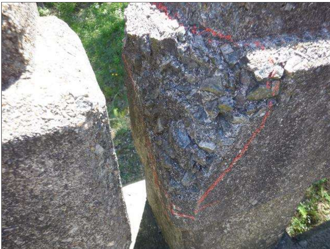
Span 1 Right Bridge Rail: 4" x 7" x 6" deep spall on concrete rail at Post 2
