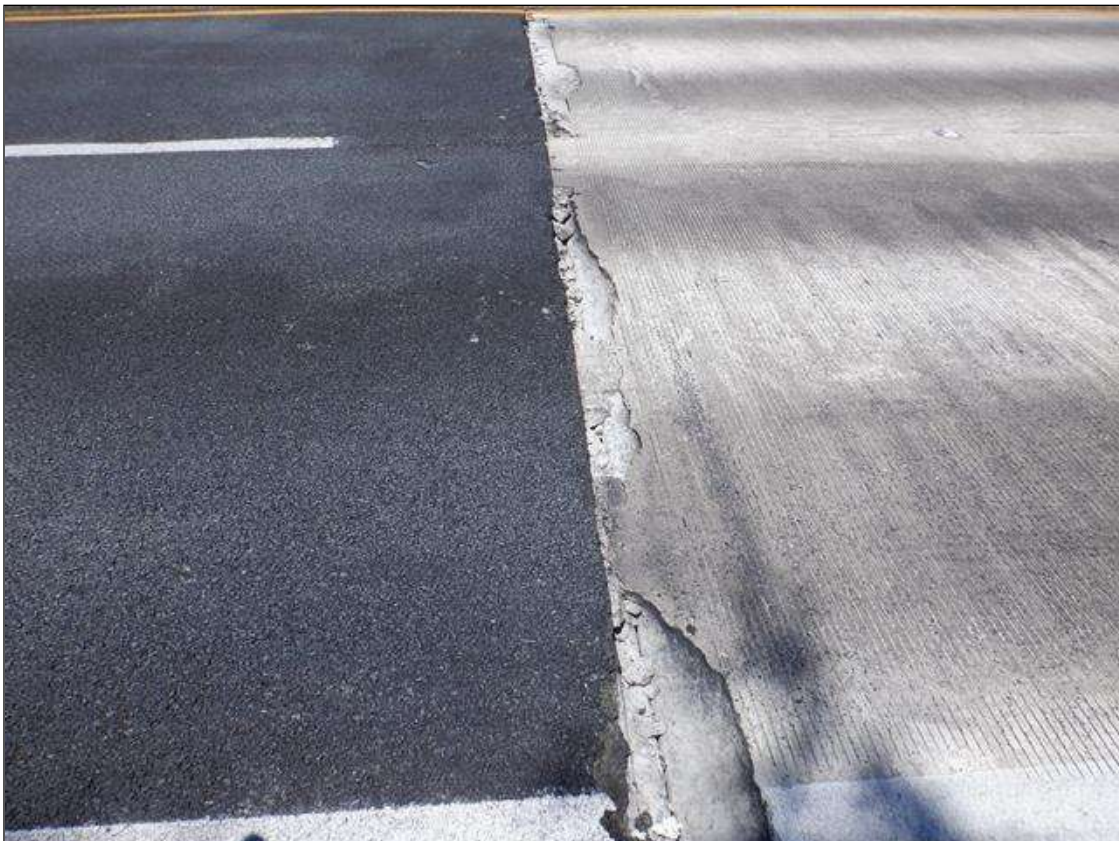
Approach 1: (3)- UP TO 11' X UP TO 1' X 3" SPALLS, AT SOUTH END.
