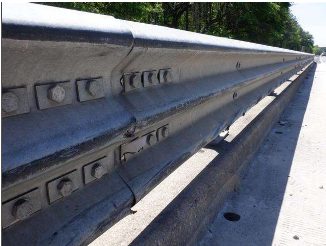
Span 2 Right Bridge Rail: (PAR) 50' OF DAMAGE TO METAL BRIDGE RAIL.
