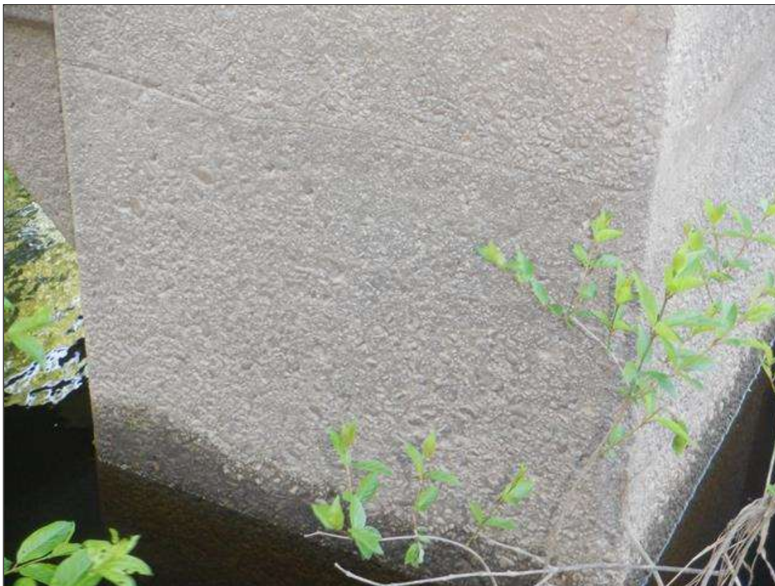
Bent 2 Pile 1: 4' ABRASION/WEAR 12' FROM BOTTOM OF CAP.
