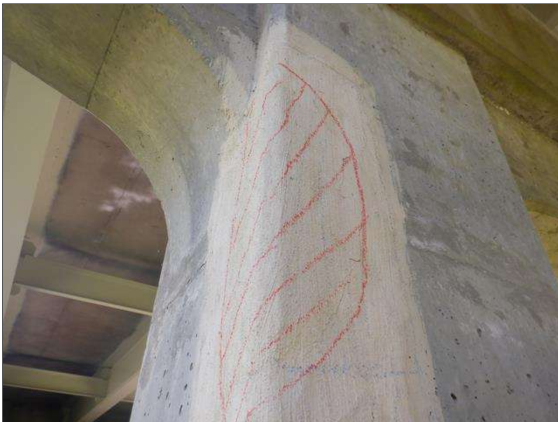
Bent 3 Pile 1: 24" x up to 7" x 4" cracked patched area and delamination, 2' from bottom of cap, on Span 3 face
