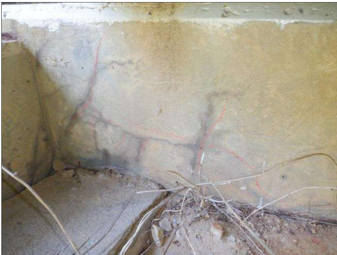
End Bent 2 Cap 1: 12' X 2' AREA OF MAP CRACKING UP TO 1/32", BEGINNING AT WEST END (PHOTO TAKEN UNDER BEAM 1).
