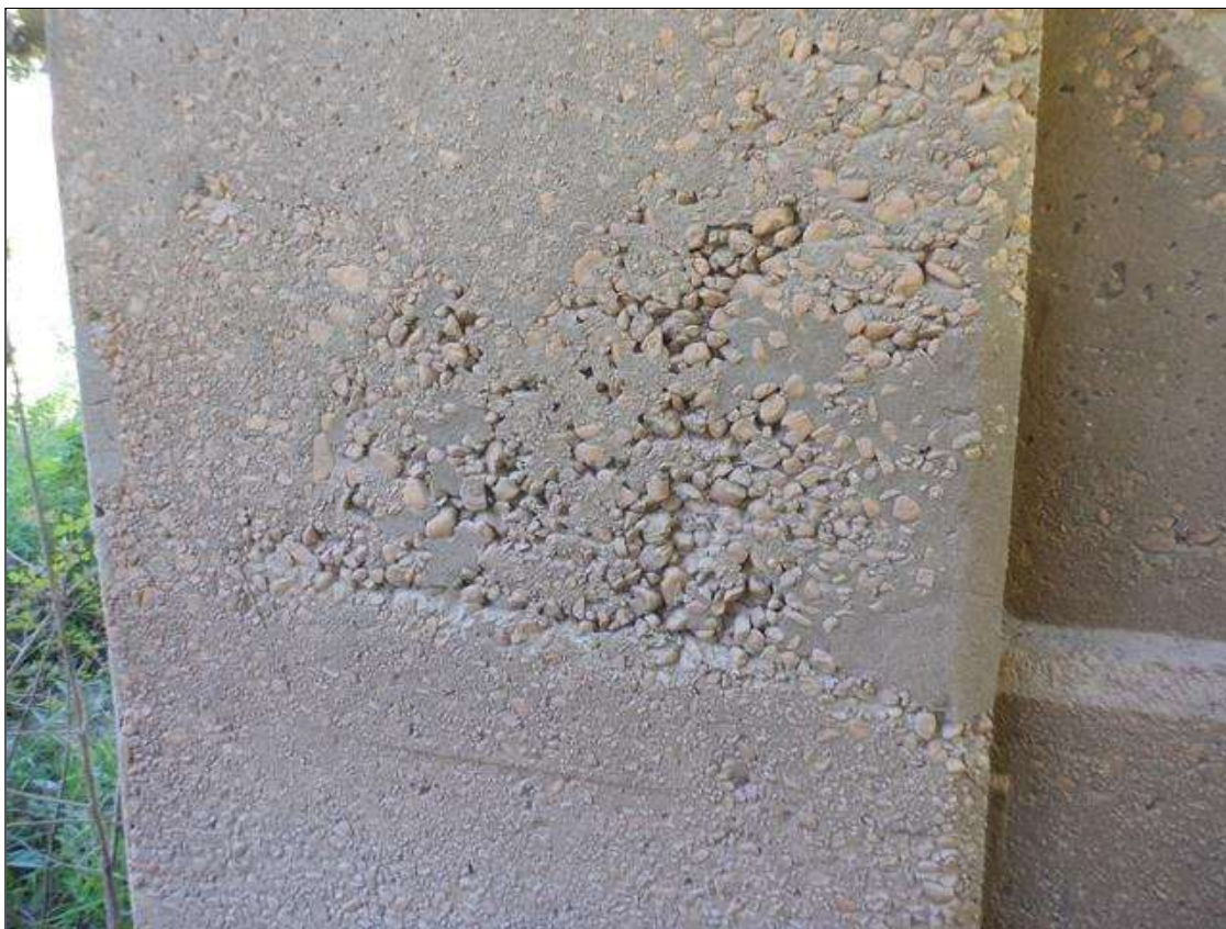
Bent 3 Pile 1: 15" x 19" area of honeycombing with loose aggregate on Span 3 face, at strut height (Span 4 face similar)
