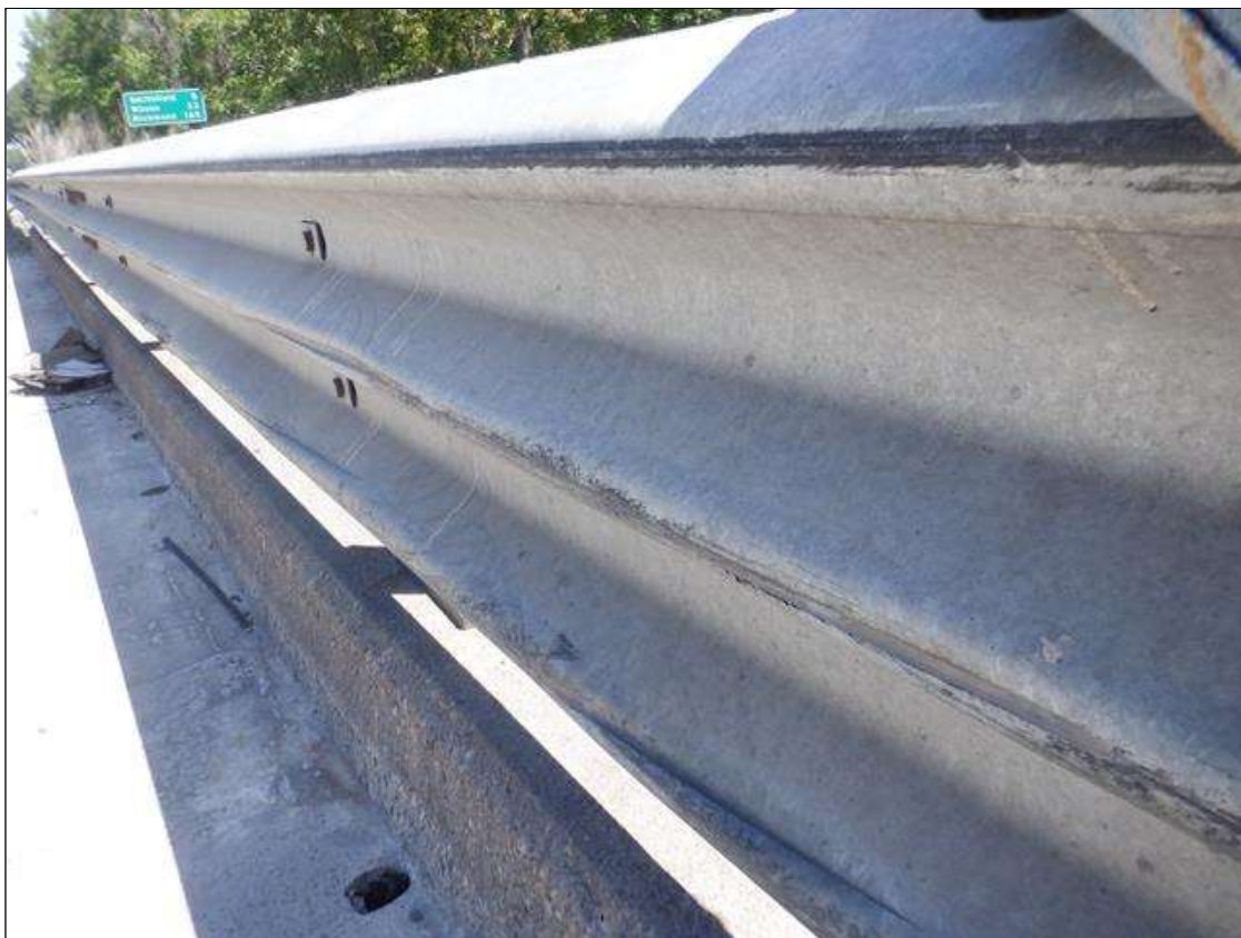
Span 4 Right Bridge Rail: 51' OF DAMAGE/SCRAPES TO METAL BRIDGE RAIL.
