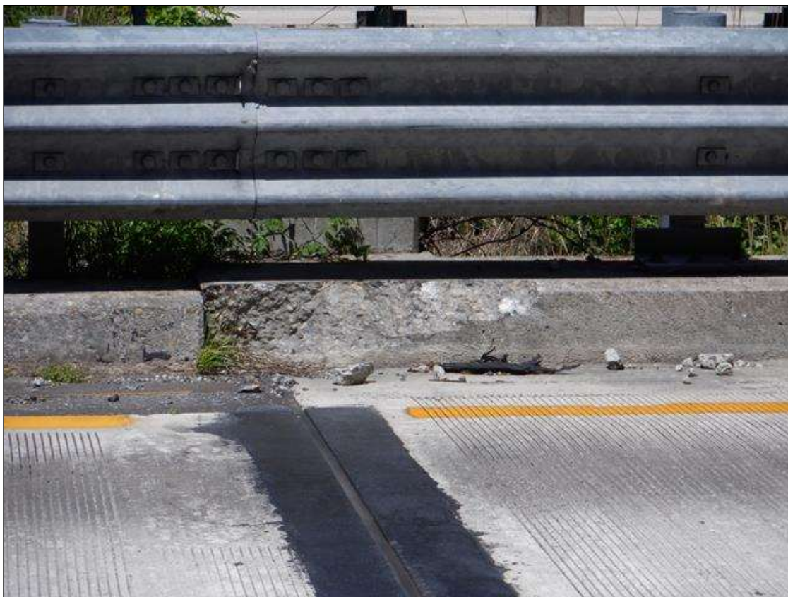
Span 1 Left Bridge Rail: 35" x 9" x 2" deep spall with exposed rebar on concrete curb at End Bent 1
