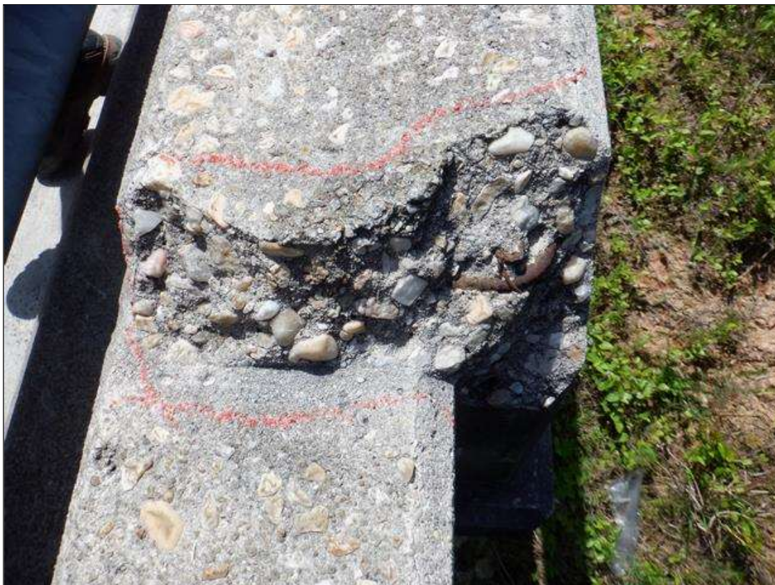
Span 1 Left Bridge Rail: 5" X UP TO 10" X 7" SPALL WITH EXPOSED REINFORCING, 18' FROM END BENT 1.
