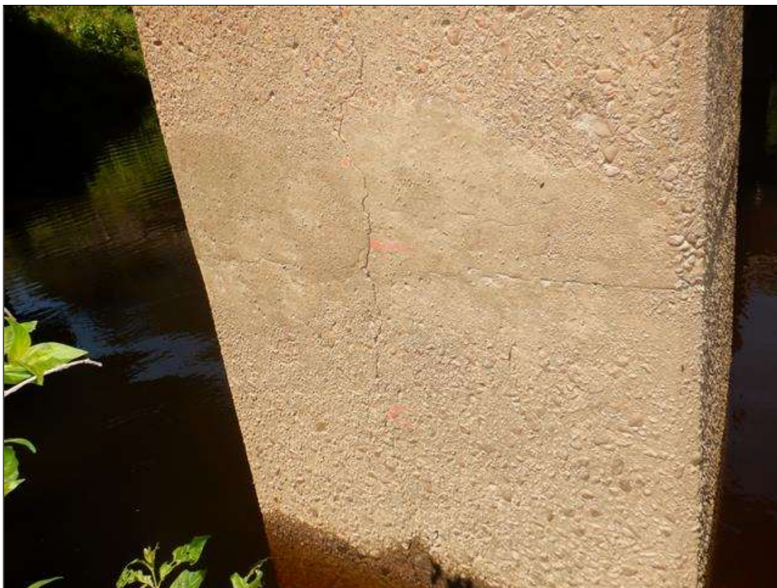
Bent 2 Pile 2: 46" x up to 1/16" vertical crack on East face, 13' from bottom of cap (Span 3 face similar)
