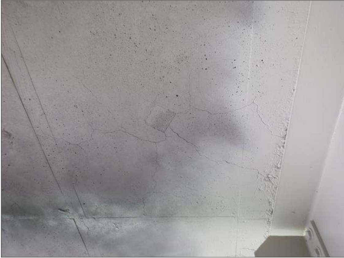
Span 4 Deck: 750 SF OF MAP CRACKING UP TO 1/32", IN UNDERSIDE OF DECK, AT RANDOM THROUGHOUT (PHOTO TAKEN BAY 2 NEAR MIDSPAN).
