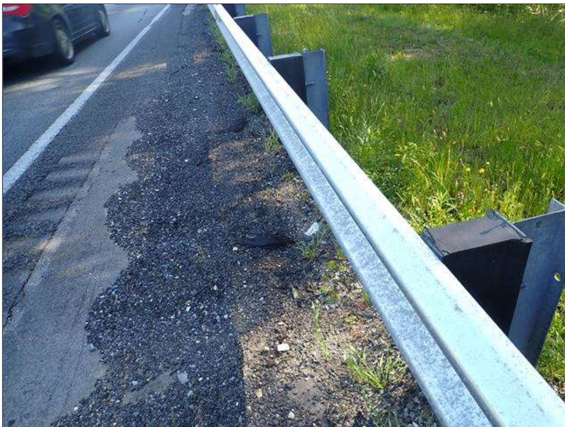
36' OF REPAIRED GUARDRAIL AT SOUTHEAST CORNER, AT END BENT 1.
