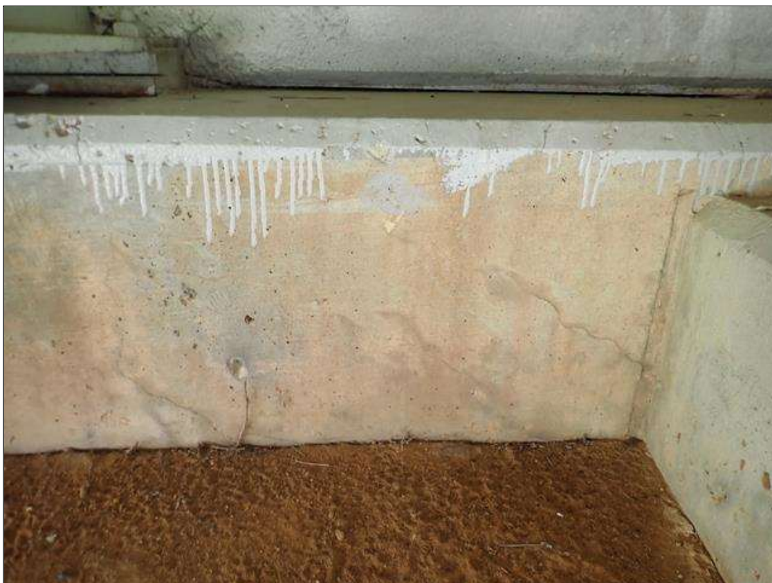
End Bent 2 Cap 1: 12' X 2' AREA OF MAP CRACKING UP TO 1/32", BEGINNING AT WEST END.
