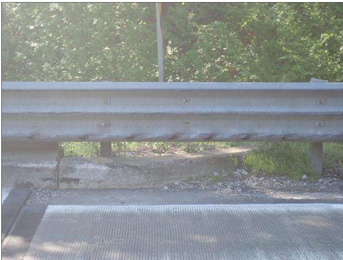
Span 1 Right Bridge Rail: 52' OF DAMAGE TO METAL BRIDGE RAIL, RAIL STILL FUNCTIONAL.
