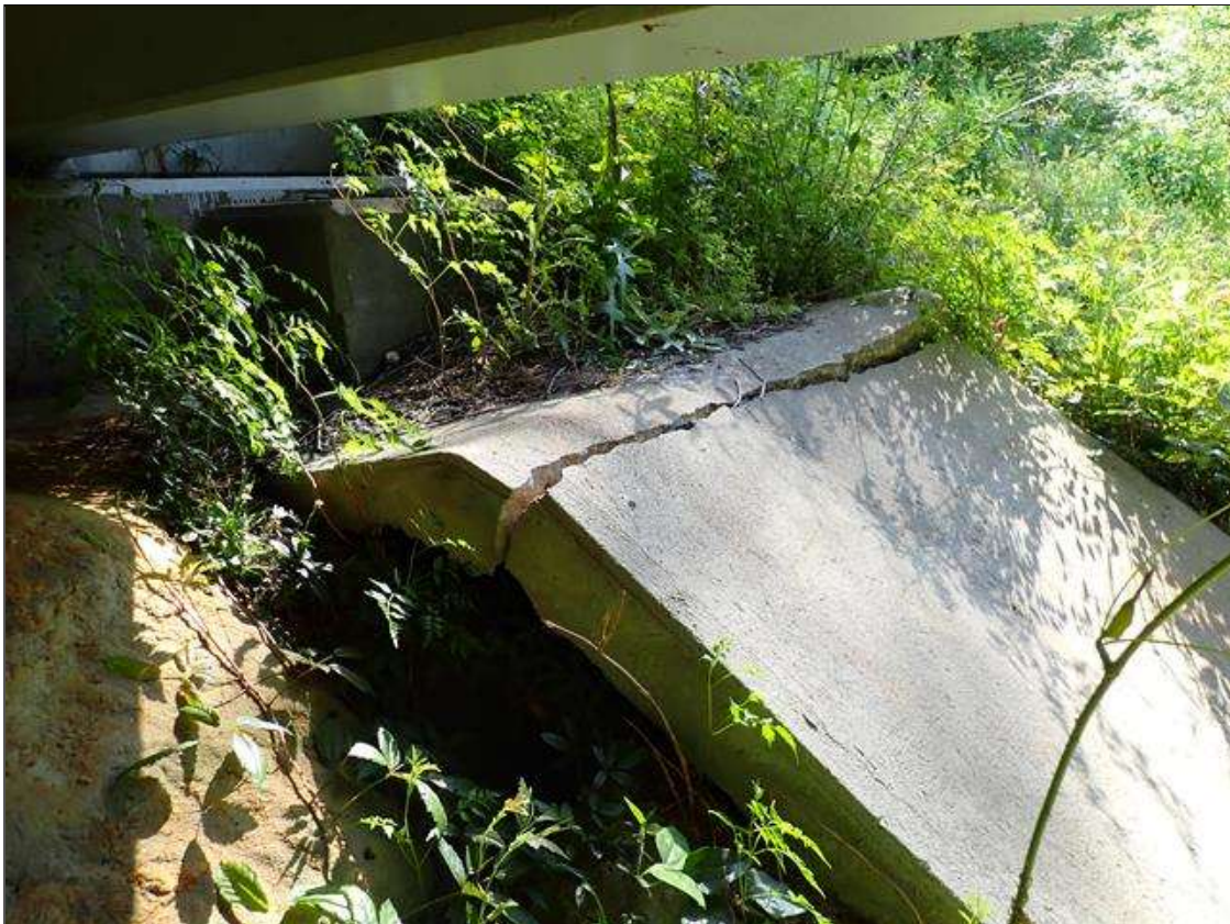
DECK DRAIN DITCH IS CRACKED AND SETTLED UP TO 6" ON EAST AND WEST SIDES OF END BENT 2.
