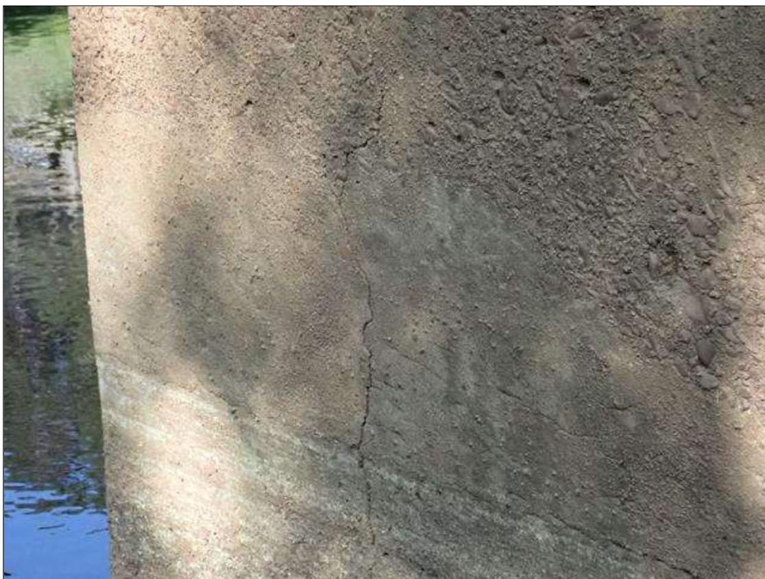
Bent 2 Pile 2: 72" x up to 1/16" vertical crack on East face, 13' from bottom of cap (Span 3 face similar)
