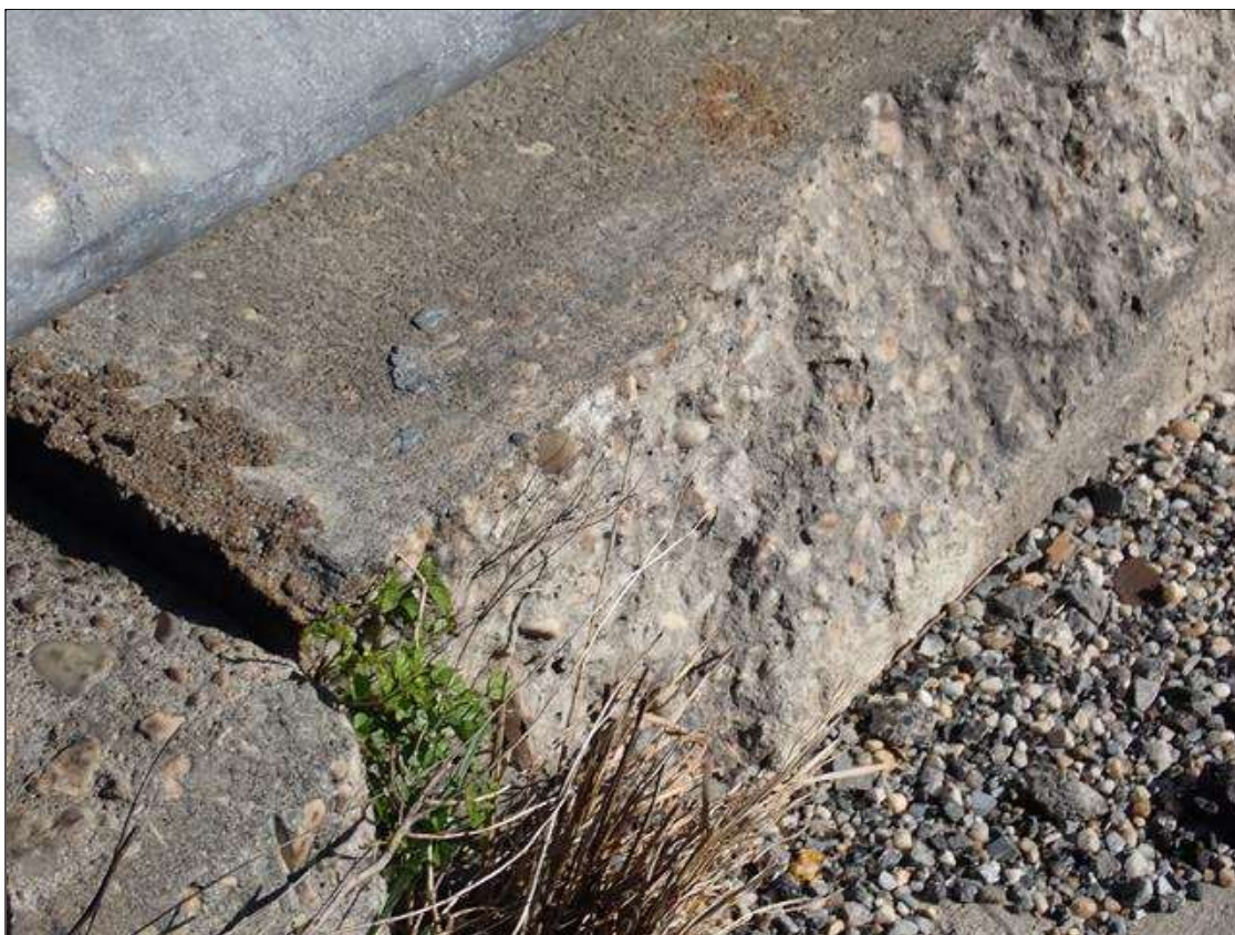
Span 1 Left Bridge Rail: 35" x 9" x 2" deep spall with exposed rebar and no measurable section loss on concrete curb at End Bent 1
