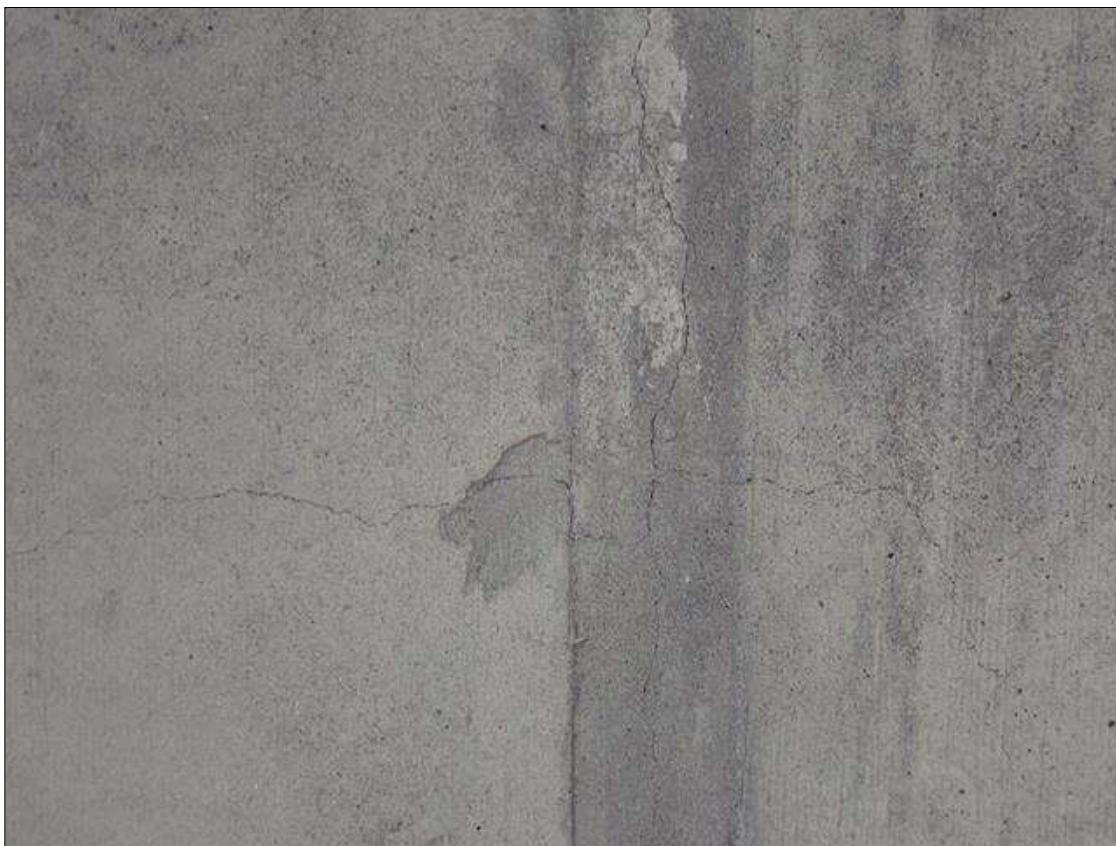
Span 1 Deck: 750 SF OF MAP CRACKING UP TO 1/32", IN UNDERSIDE OF DECK, AT RANDOM THROUGHOUT.
