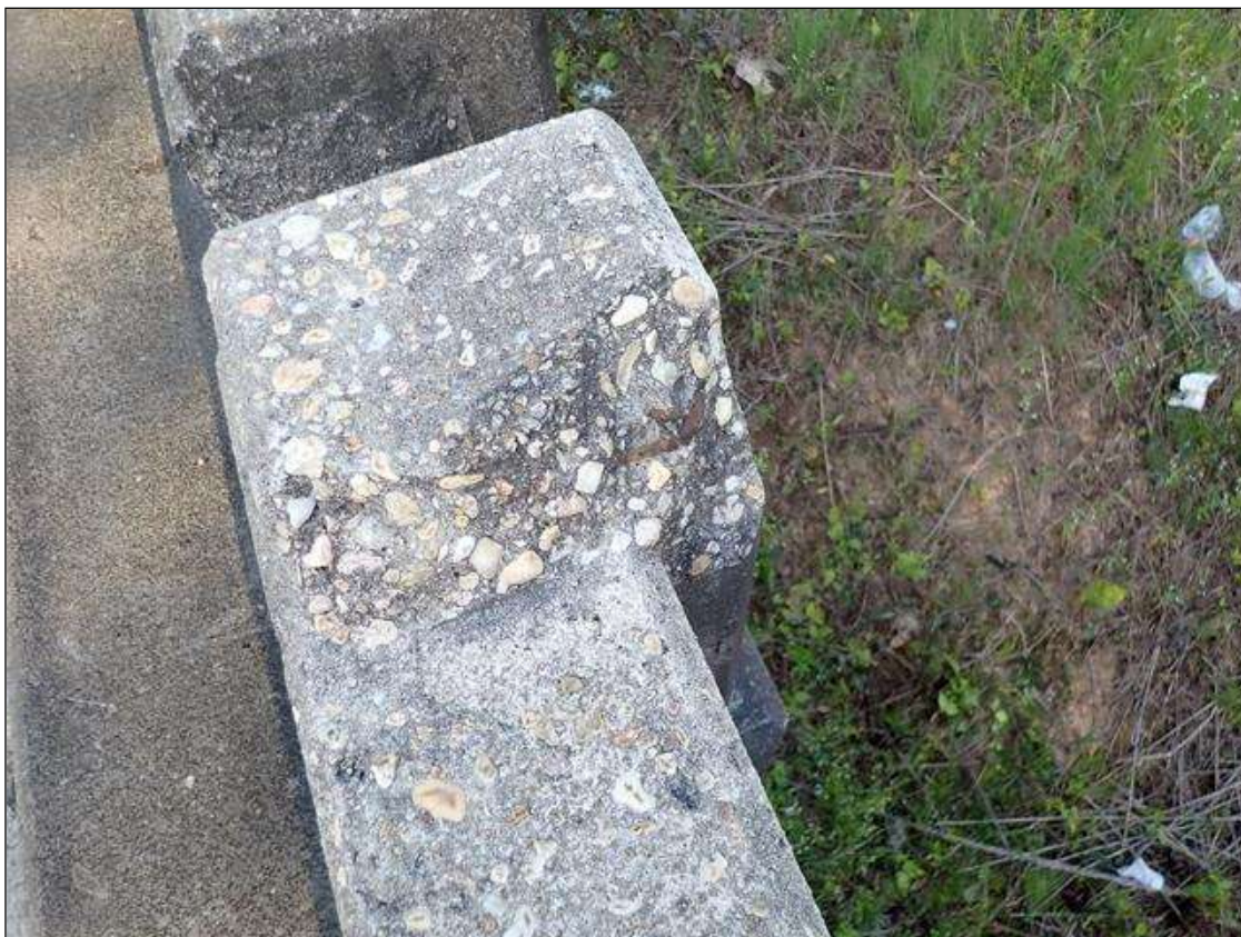
Span 1 Left Bridge Rail: (2)- UP TO 4" X 10" X 7" SPALLS WITH EXPOSED REBAR, NO MEASURABLE SECTION LOSS, IN TOP OF POSTS, 17' FROM END BENT 1.
