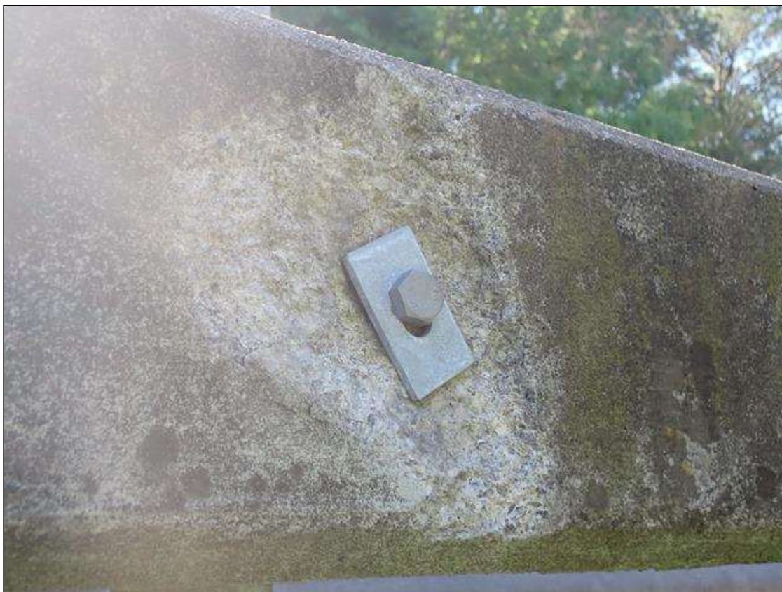
Span 1 Left Bridge Rail: (5) up to 7" x 9" x 1" deep spalls on outside face of concrete rail at bolt locations, no exposed rebar.
