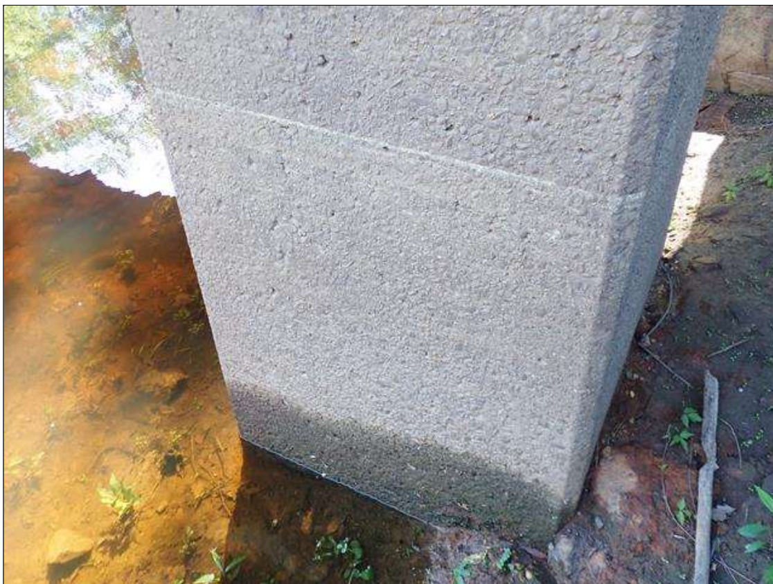
Bent 1 Pile 1: 2' ABRASION/WEAR 12' FROM BOTTOM OF CAP WITH AGGREGATE INTACT
