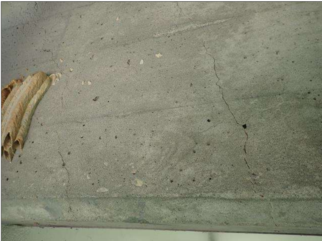
Span 4 Beam 1: 5 FULL HEIGHT HAIRLINE VERTICAL CRACKS IN BAY 1 END BENT DIAPHRAGM.
