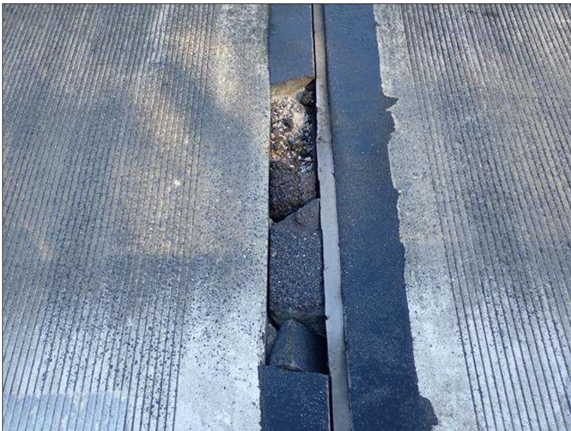
Span 2 Expansion Joint at Bent 1: 32" x 6" x 3" deep spall in the right Northbound lane joint header, no exposed rebar.
