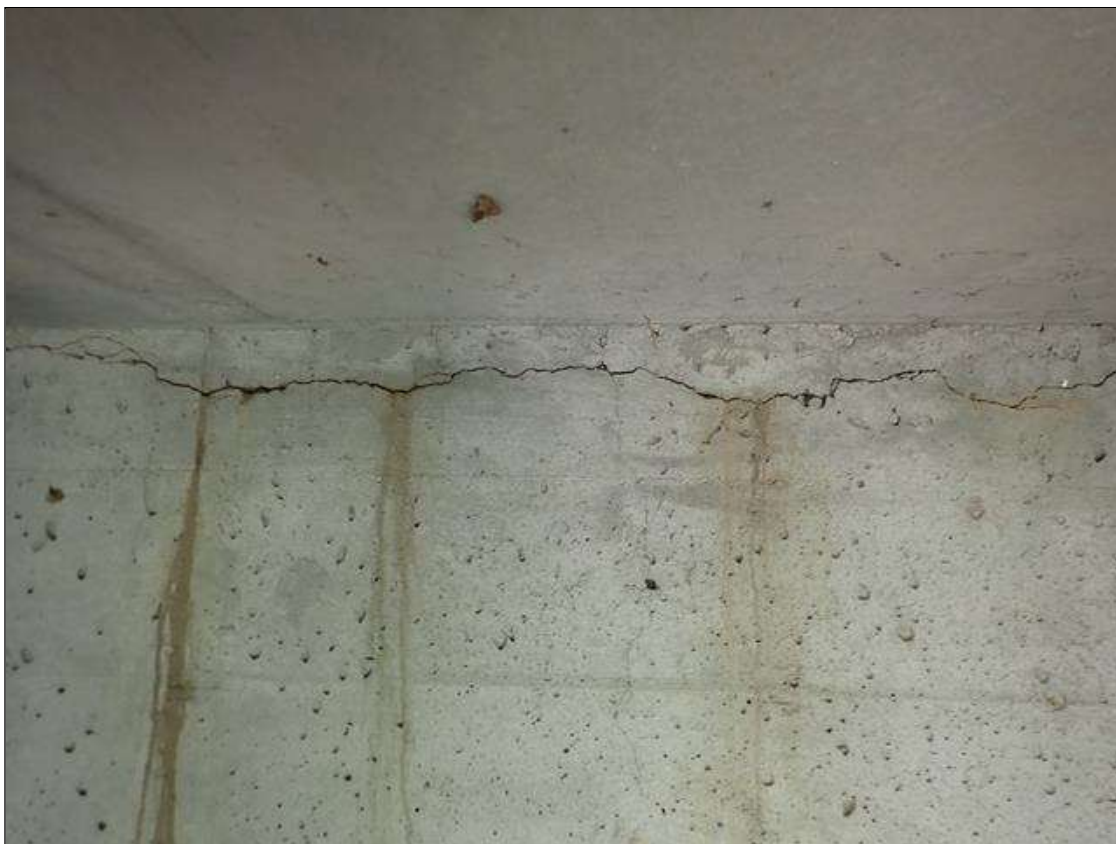
End Bent 2 Abutment: HORIZONTAL AND VERTICAL CRACKS UP TO 1/8", SOME WITH EFFLORESCENCE, IN ALL BAYS.
