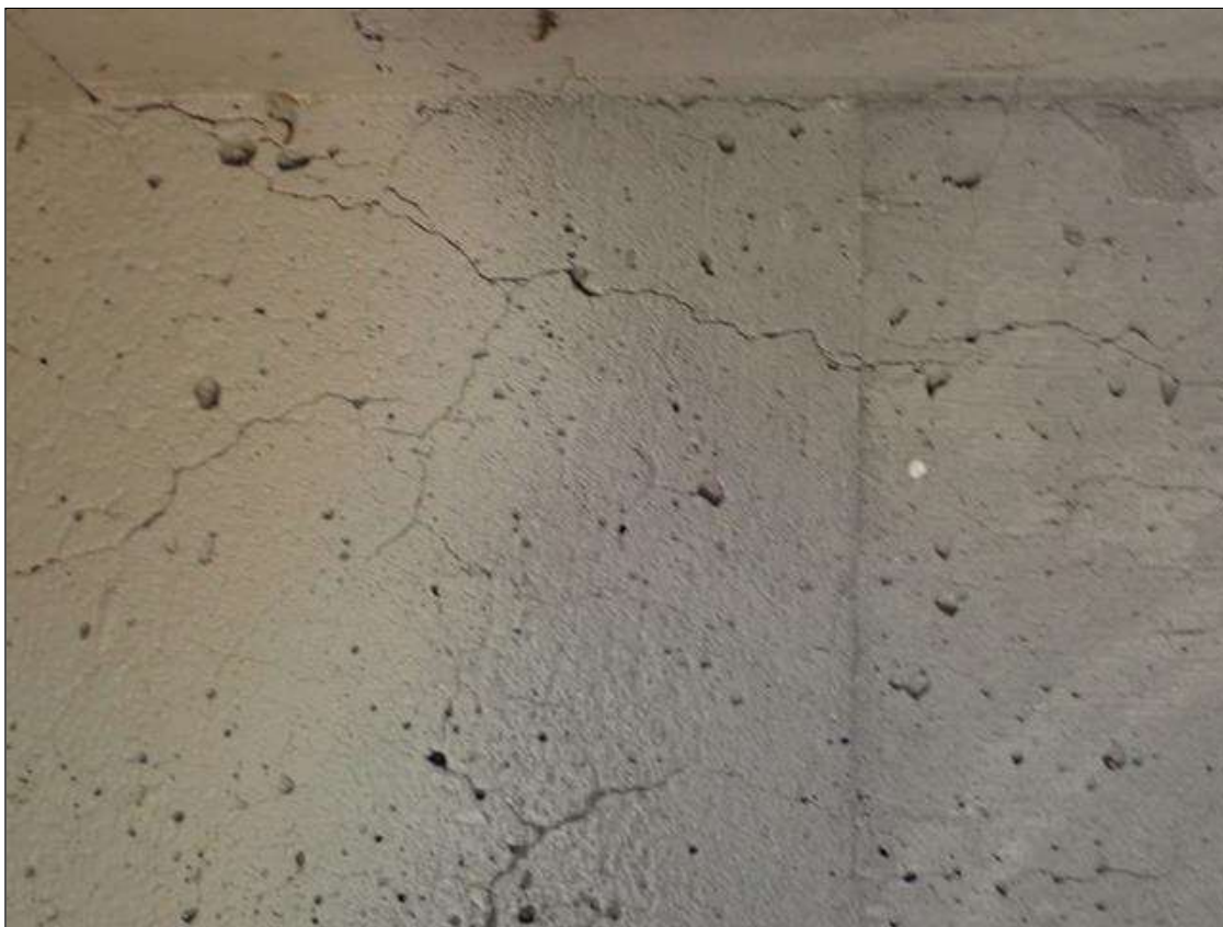
End Bent 1 Abutment: 32' OF HORIZONTAL AND VERTICAL CRACKS UP TO 1/32", SOME WITH EFFLORESCENCE.
