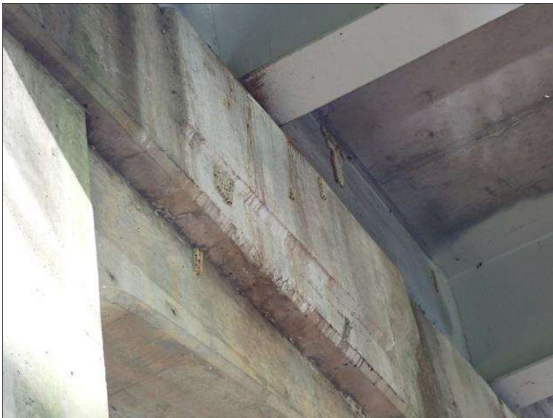
Bent 1 Cap 1: 6' X UP TO 16" SOUND PATCHED AREA, NORTH FACE, UNDER BEAM 3.
