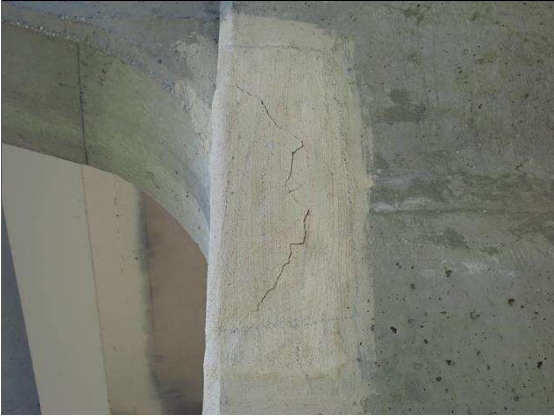
Bent 3 Pile 1: 24" x up to 7" x 4" cracked patched area and delamination, 2' from bottom of cap, on Span 3 face
