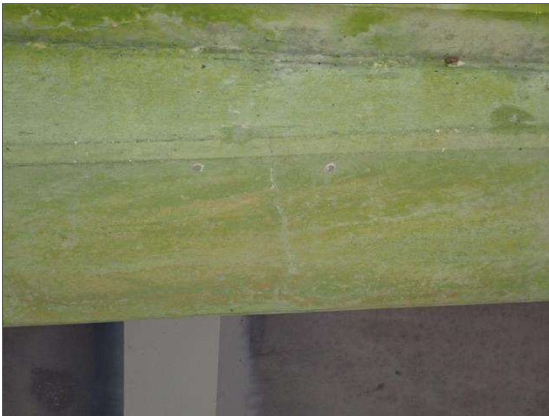
Bent 2 Cap 1: (3) up to 20" x 1/64" transverse cracks, some with efflorescence, on bottom of corbel between Columns 1 and 2
