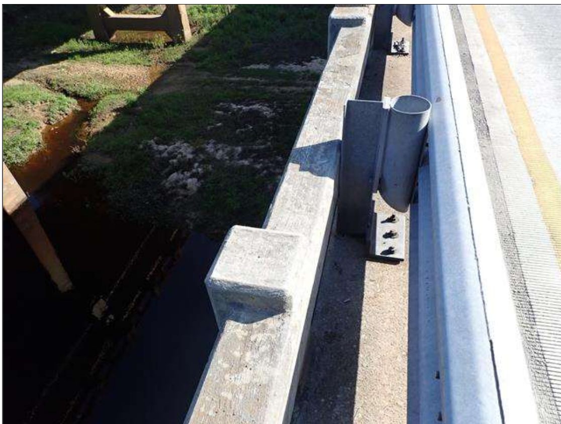
Span 2 Left Bridge Rail: 10' repaired section of concrete rail at midspan
