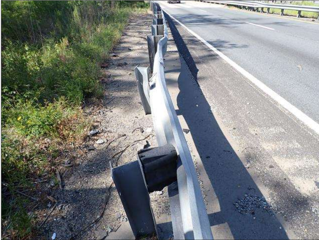
15' LONG SECTION OF IMPACT DAMAGE TO APPROACH GUARDRAIL ON NORTHEAST CORNER 50' FROM BRIDGE, RAIL STILL FUNCTIONAL.
