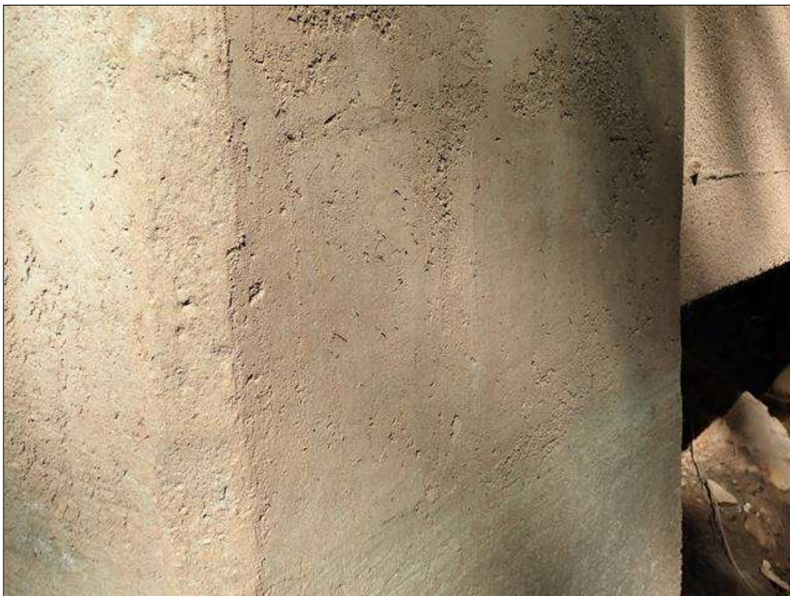
Bent 1 Pile 2: 2' diameter area of sound patch on Span 2 face, 12' from bottom of cap.
