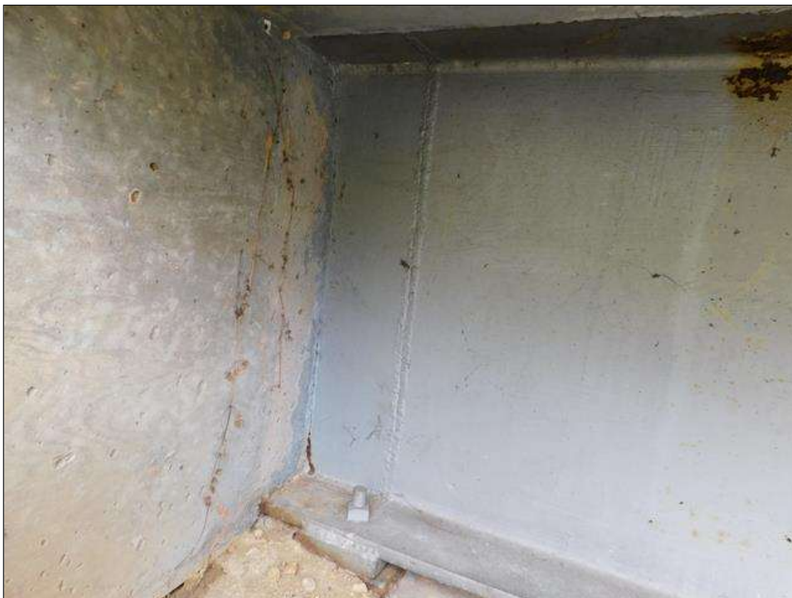
Span 1 Beam 1: Temporary Repair - 7" x 31" area of replaced beam at End Bent 1
