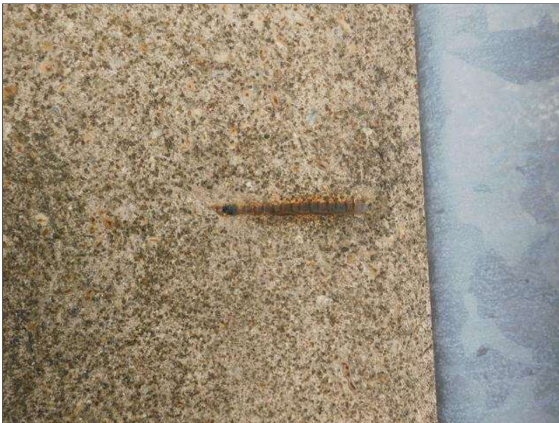
Span 4 Left Bridge Rail: 6" x 1" x 1/2" deep spall with exposed rebar on top of curb, 7' from Bent 3
