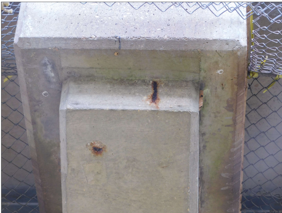
Bent 3 Cap 1: (2) up to 3" x 6" x 1" deep spall with exposed rebar on West face of corbel
