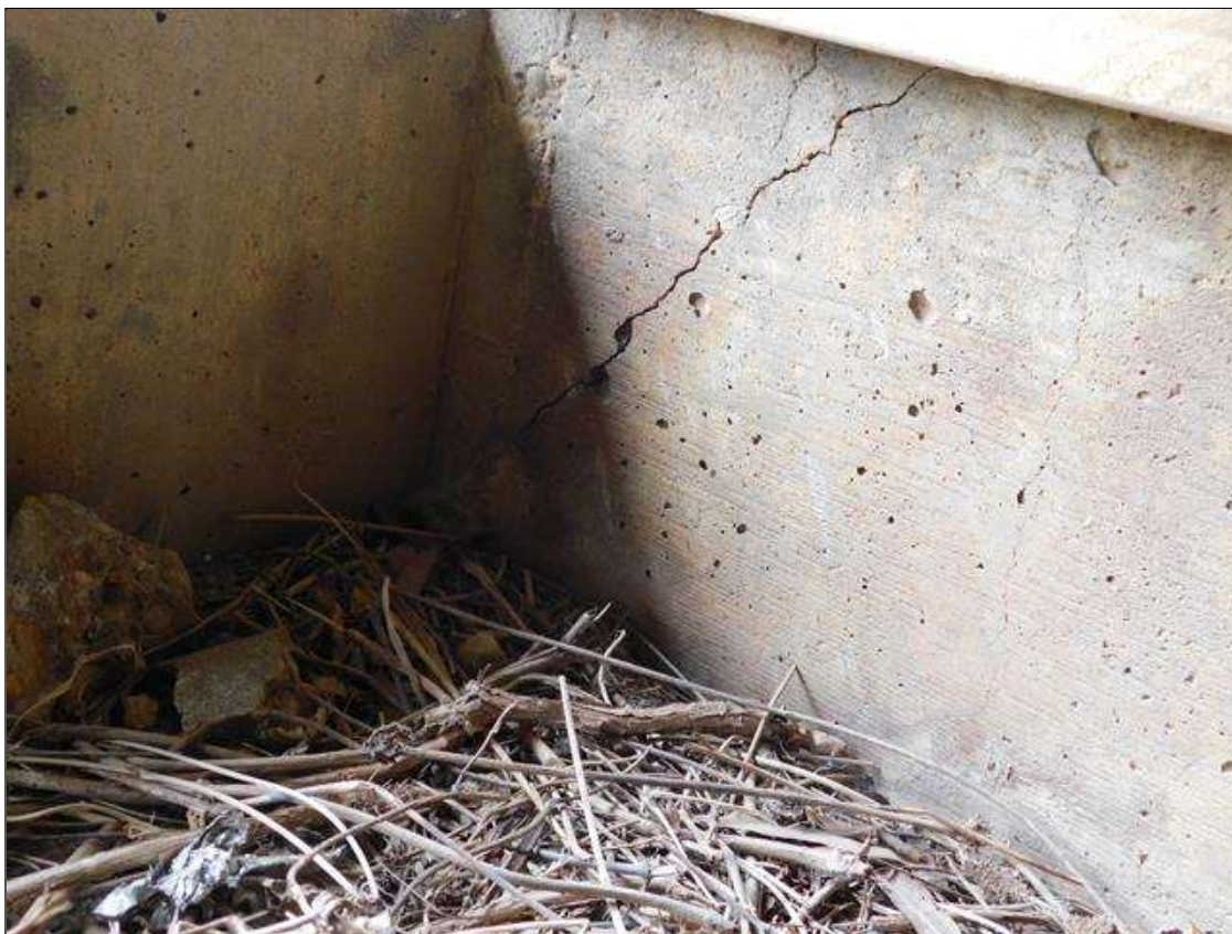
End Bent 1 Cap 1: 16" up to 1/16" diagonal crack under Beam 4
