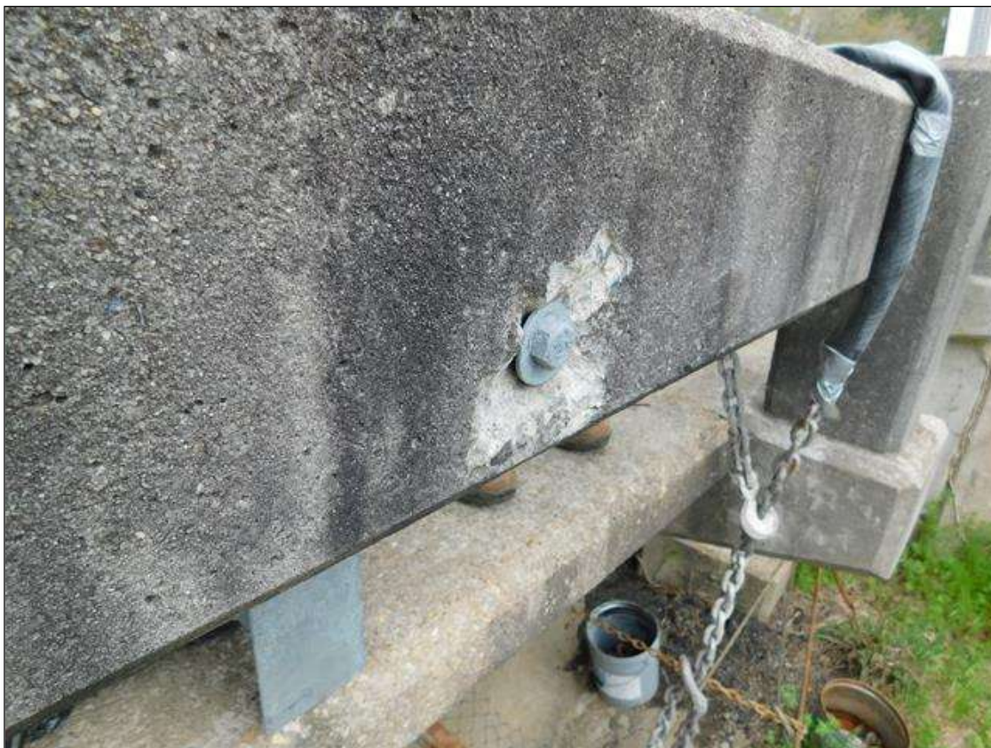
Span 4 Right Bridge Rail: 5" x 4" x 1/2" deep spall on outside face of concrete rail
