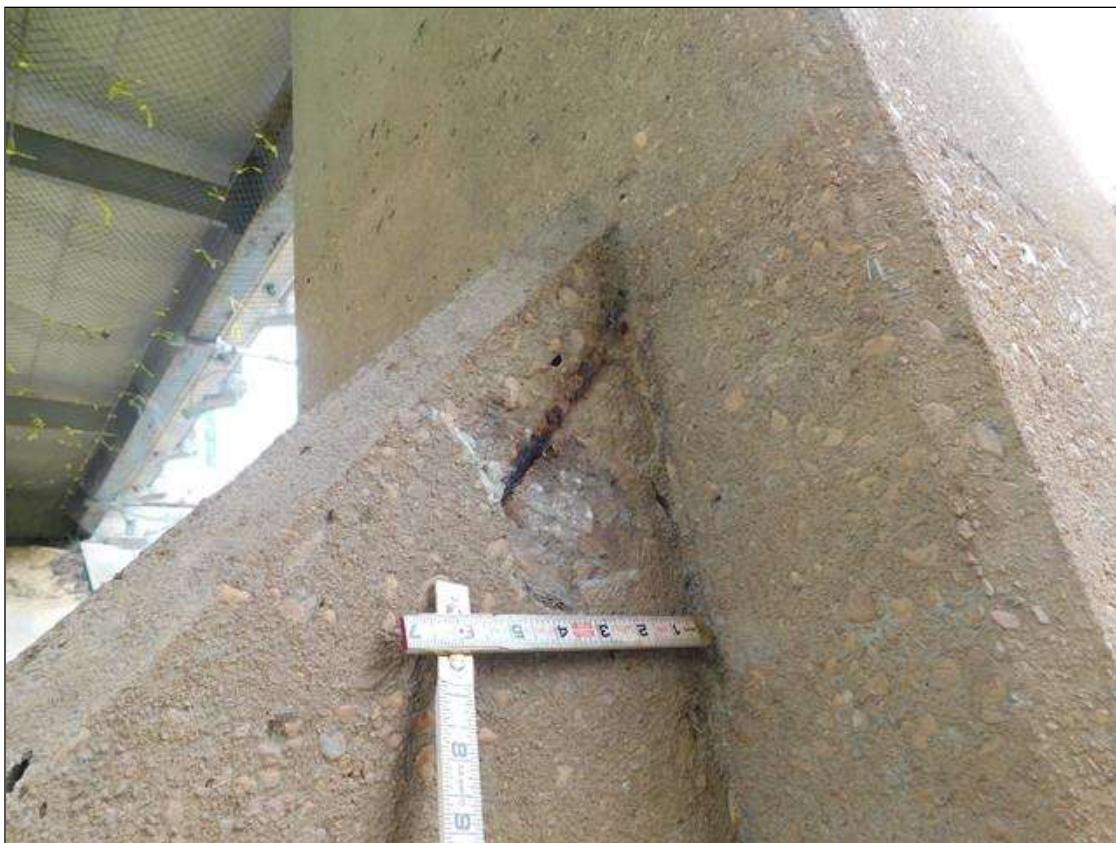
Bent 3 Pile 2: 6" x 8" x 1" deep spall with exposed rebar on Span 3 face of corbel above strut
