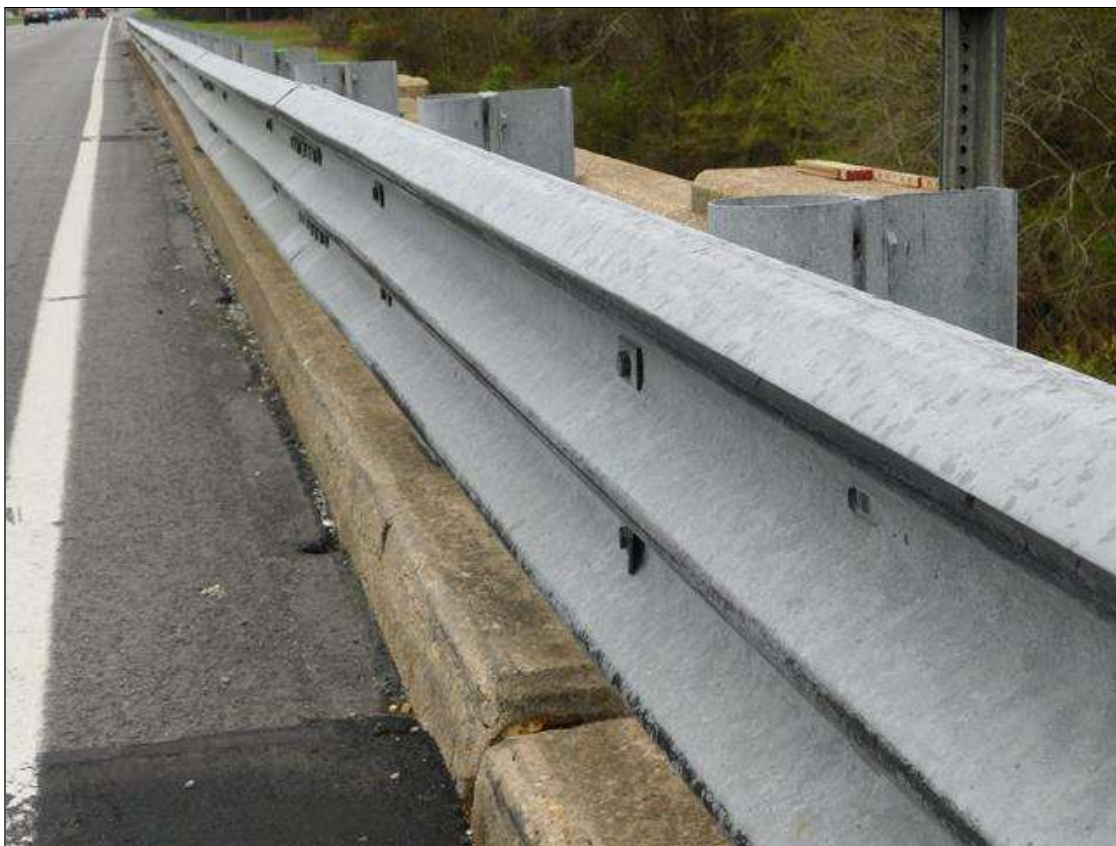
Span 4 Left Bridge Rail: 22' scrapes on metal rail at End Bent 2
