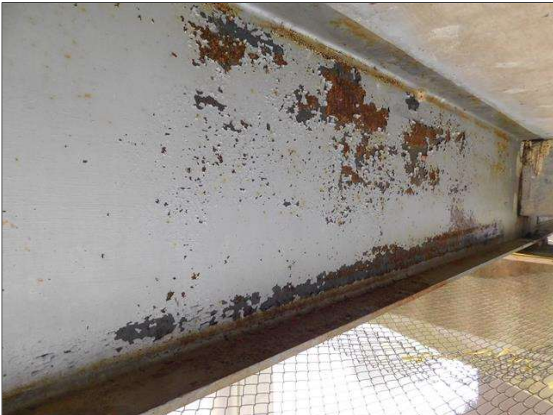
Span 1 Beam 2: 48' peeling paint with rust on web
