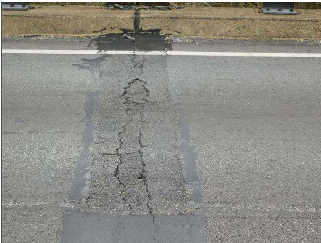
Expansion Joint: 14' x 1' area of up to 1/8" transverse cracks in East lane
