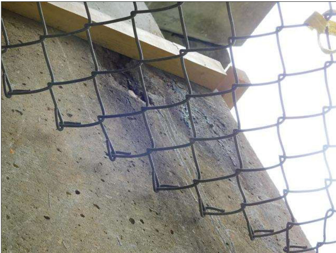
Bent 3 Cap 1: 4" x 6" x 1" deep spall with exposed rebar on Span 3 face at East end
