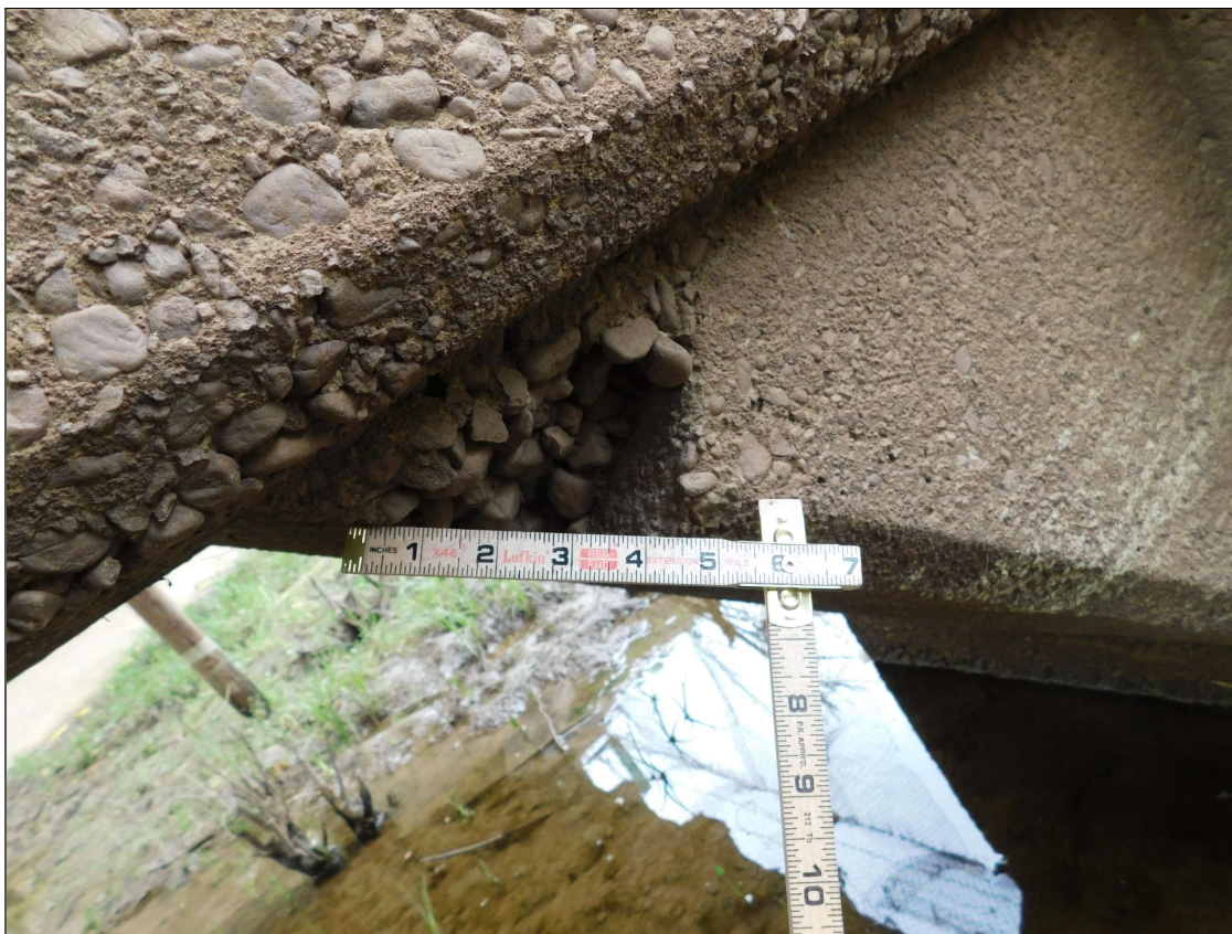
Bent 3 Pile 2: 4" x 4" x 3" deep spall on Span 3 face of corbel under strut
