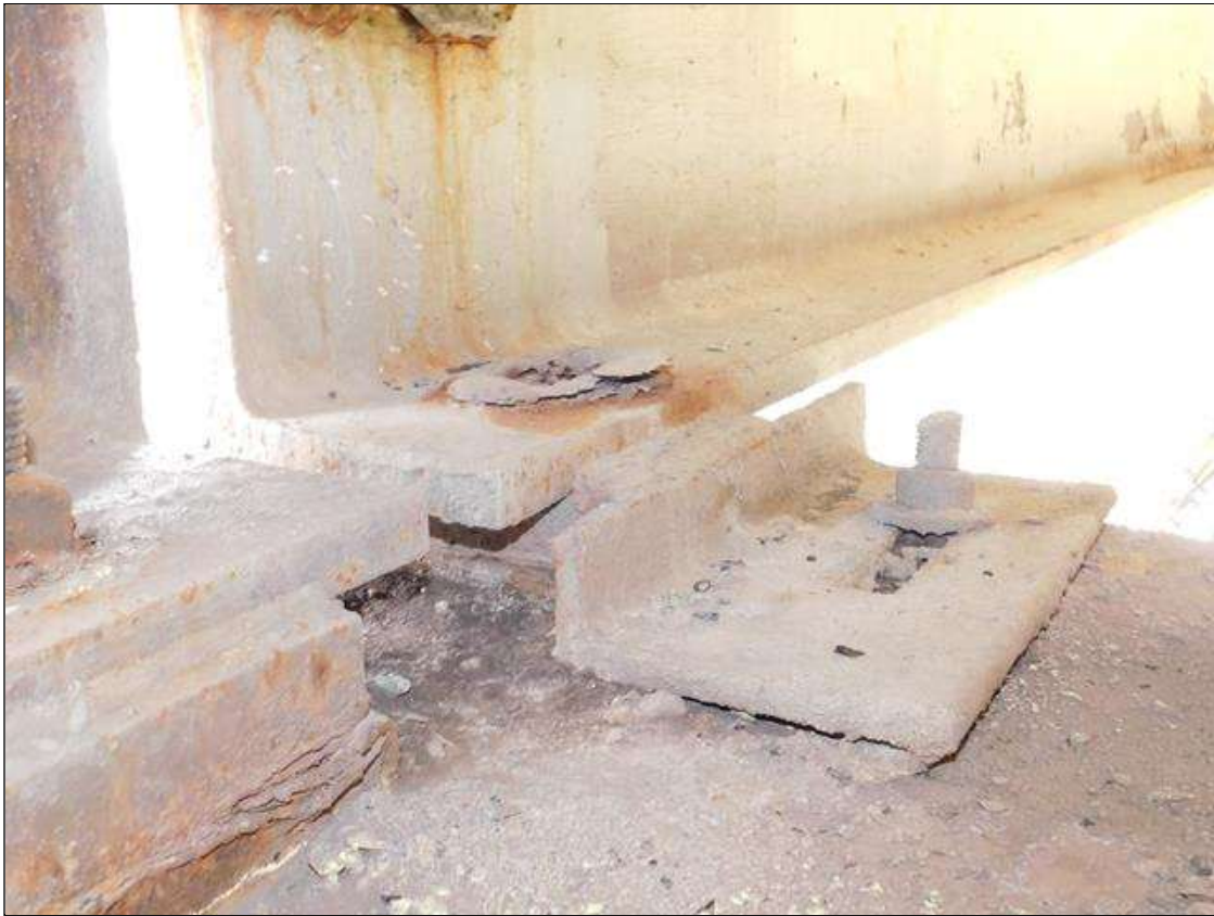
Span 3 Beam 4 Far Bearing: Temporary repair - Plate bolted on left side of bearing
