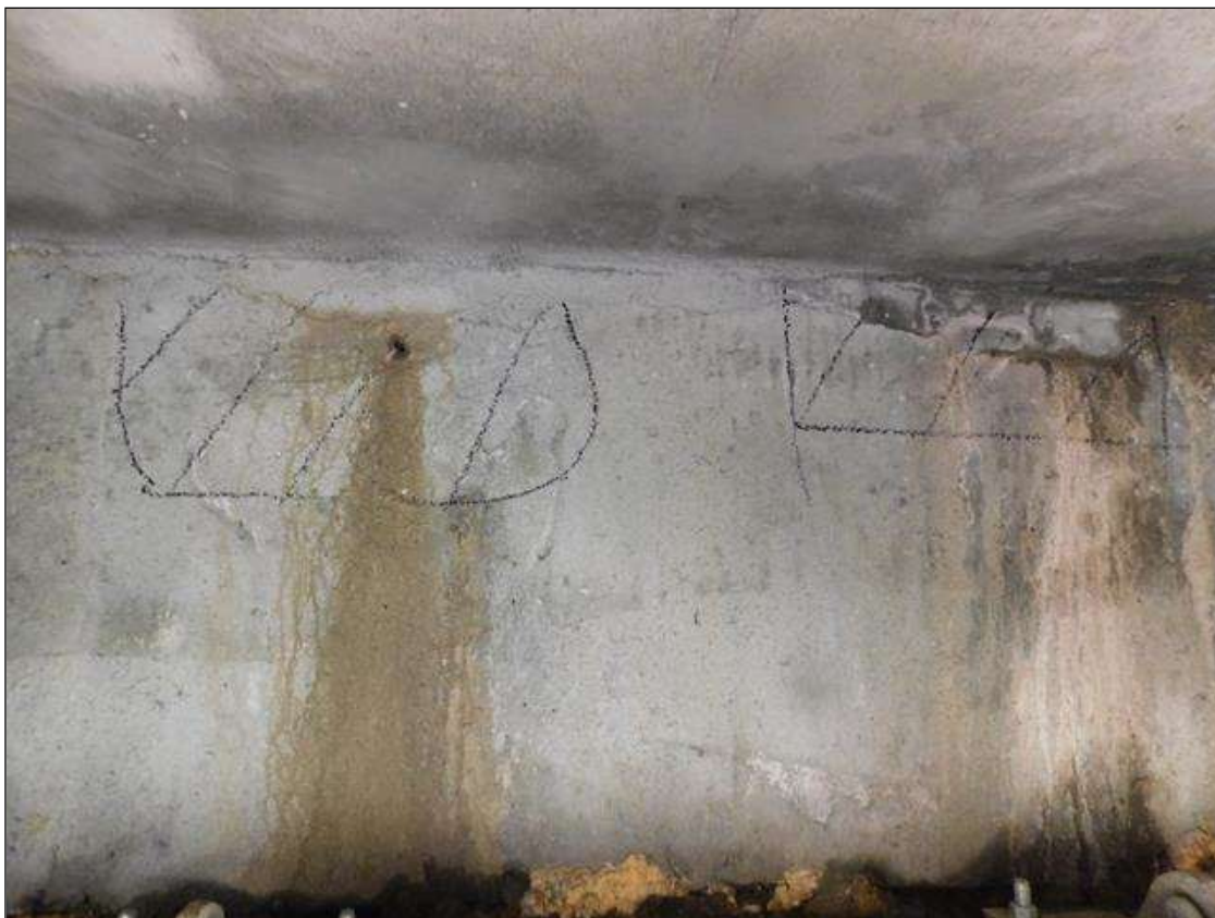
End Bent 2 Abutment/Backwall : (2) up to 24" x 12" area of delamination in Bay 1
