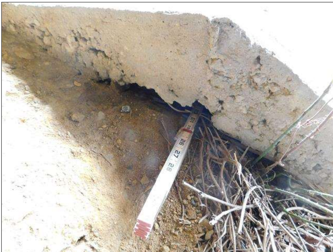
12" x 3" area of up to 24" undermining under End Bent 2 slope protection at East end (West end similar)
