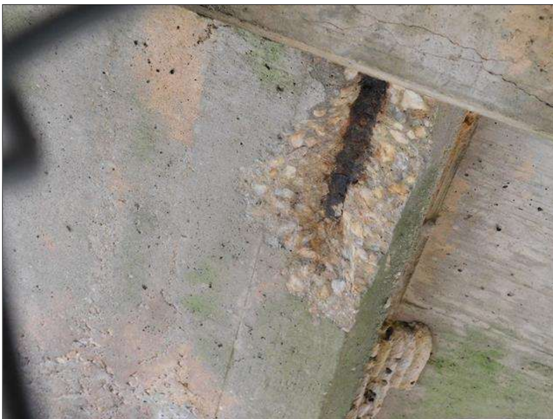
Bent 1 Pile 1: 12" x 5" x 1" deep spall with exposed rebar on Span 1 face (PM)
