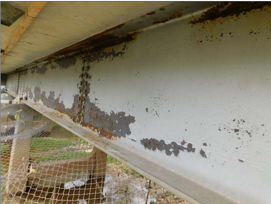
Span 4 Beam 4: Full length peeling paint with rust on both flanges and web
