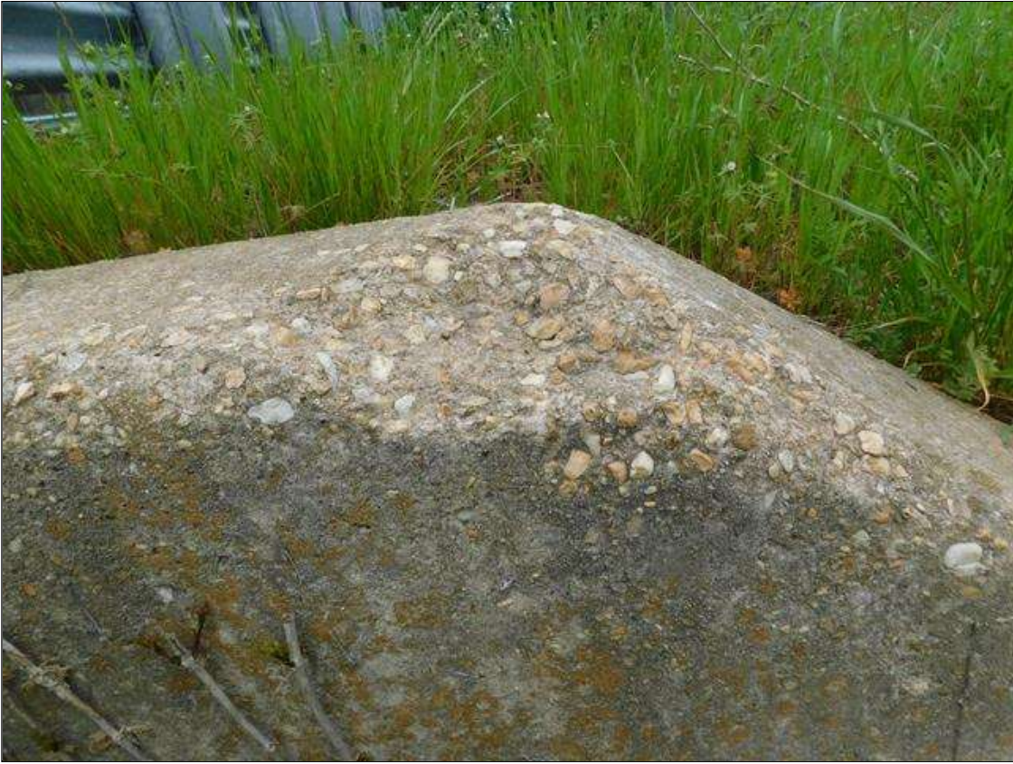
24" x 12" x 2" deep spall on Northwest wingwall
