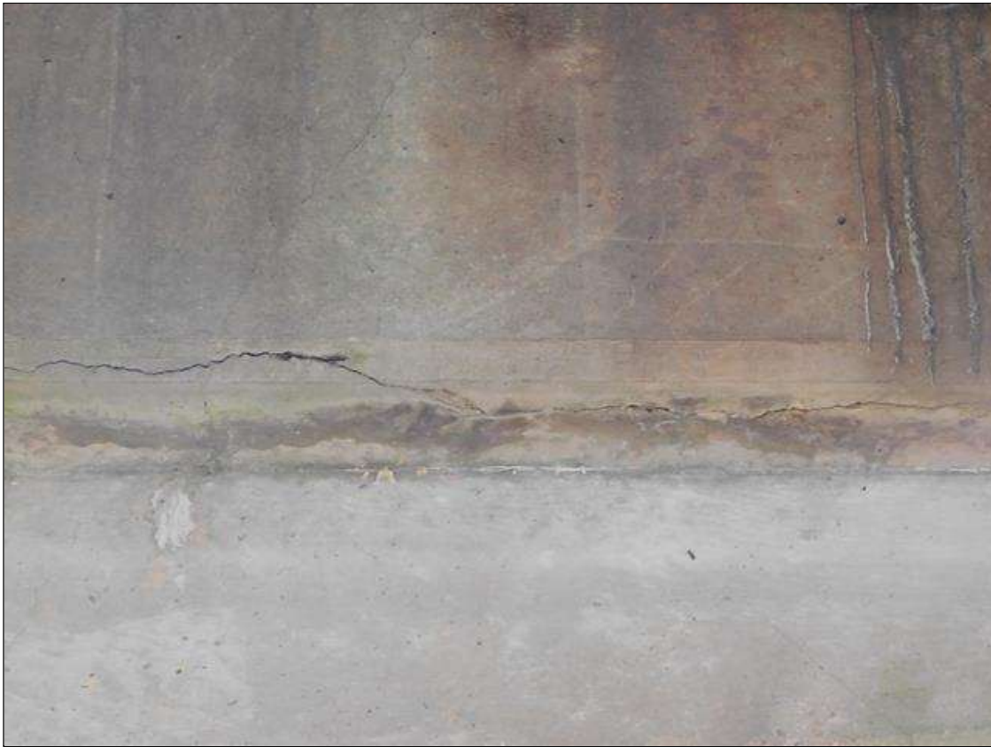
Bent 3 Cap 1: 30" up to 1/16" horizontal crack on Span 3 face
