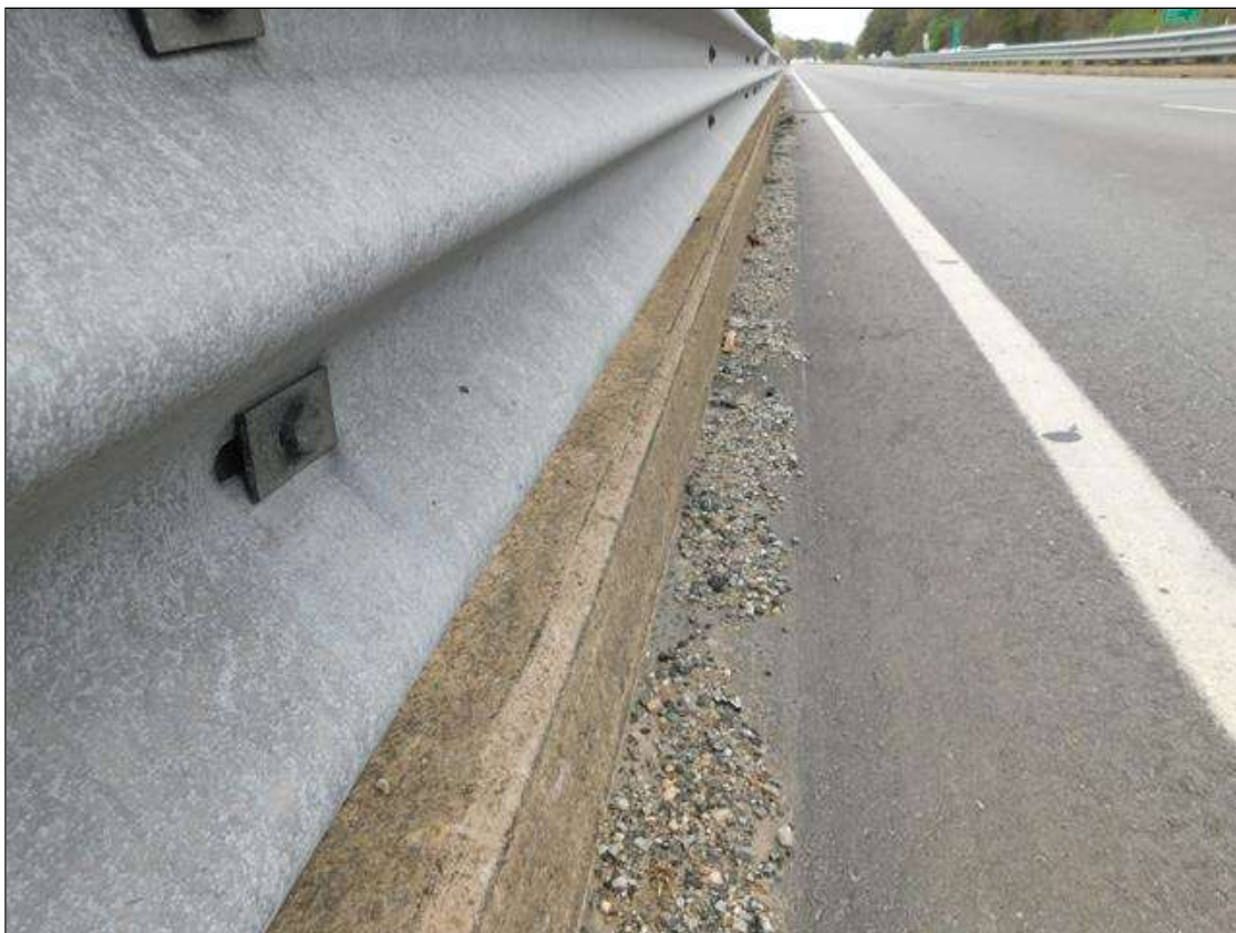
Full length x 1' dirt and debris in West gutter
