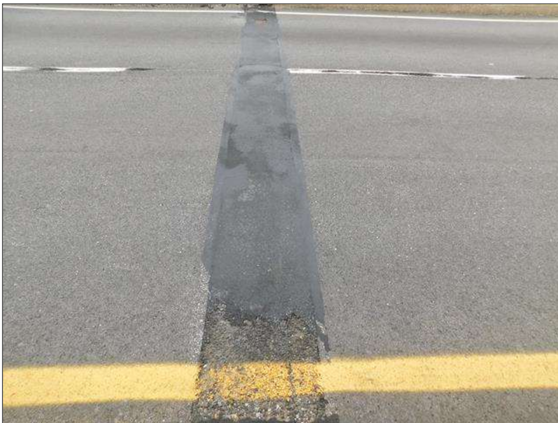
Expansion Joint : (2) up to 20" x 20" x 1/2" deep area of missing asphalt wearing surface along joint
