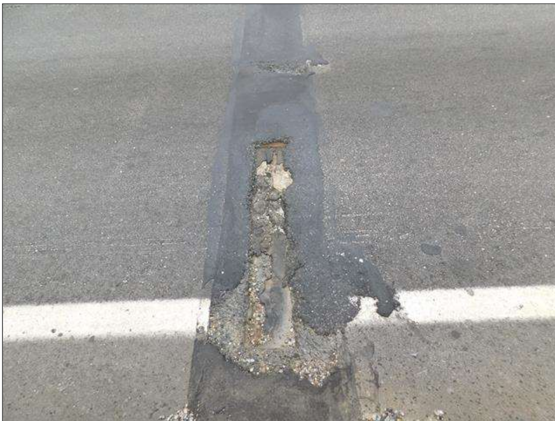
Expansion Joint : (2) up to 36" x 7" x 1" deep area of missing asphalt wearing surface along joint
