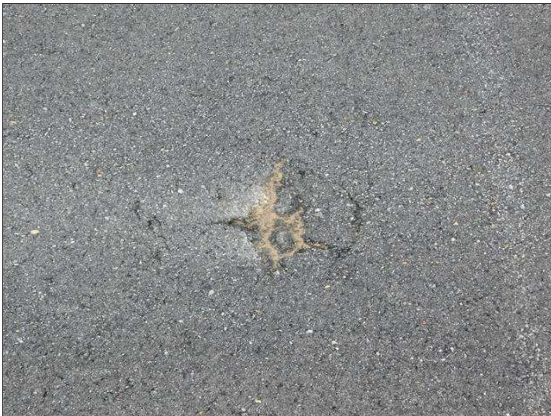
Span 3 Wearing Surface: 6" x 6" area of hairline longitudinal and transverse cracks in East lane, 9' from Bent 2
