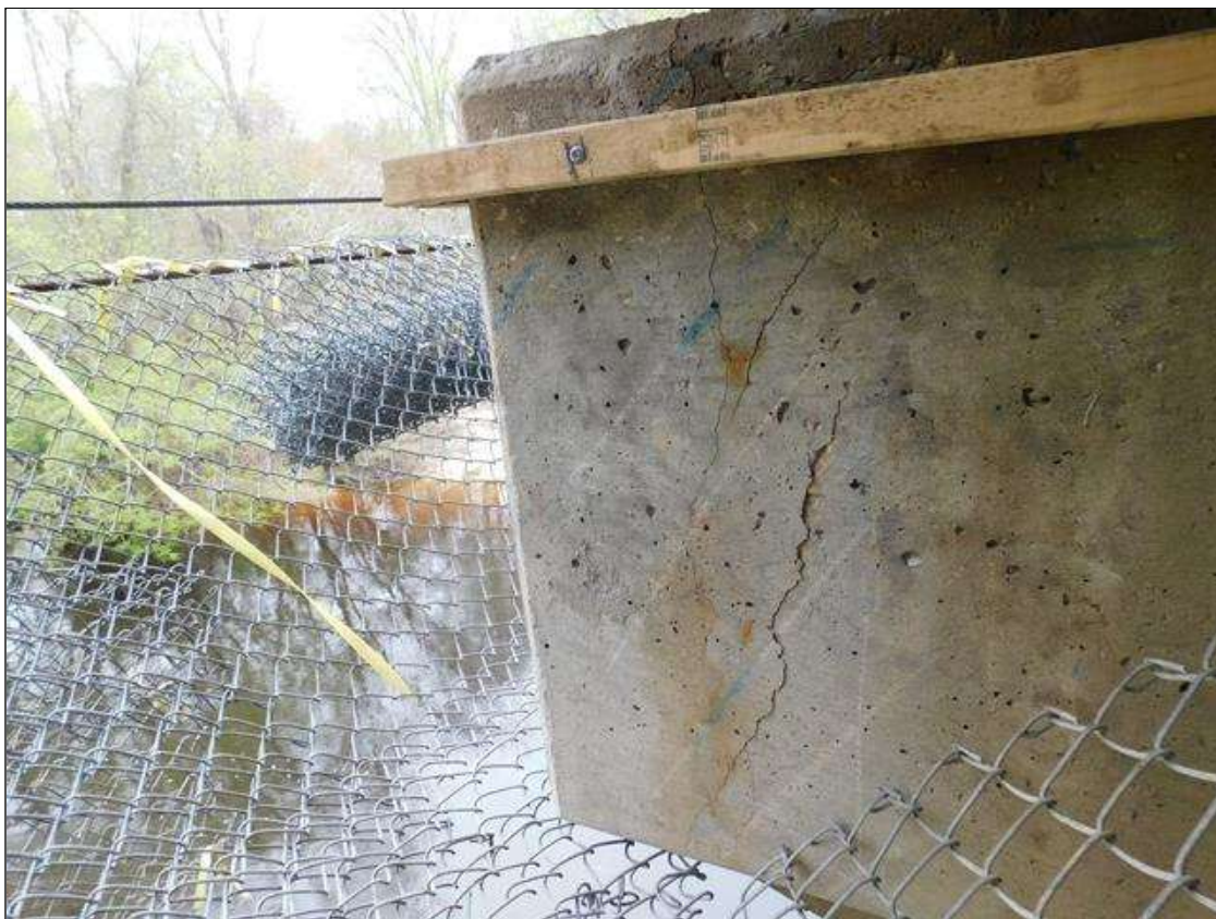
Bent 1 Cap 1: 12" x 24" area of delamination with hairline vertical, diagonal cracks on Span 1 face at West end
