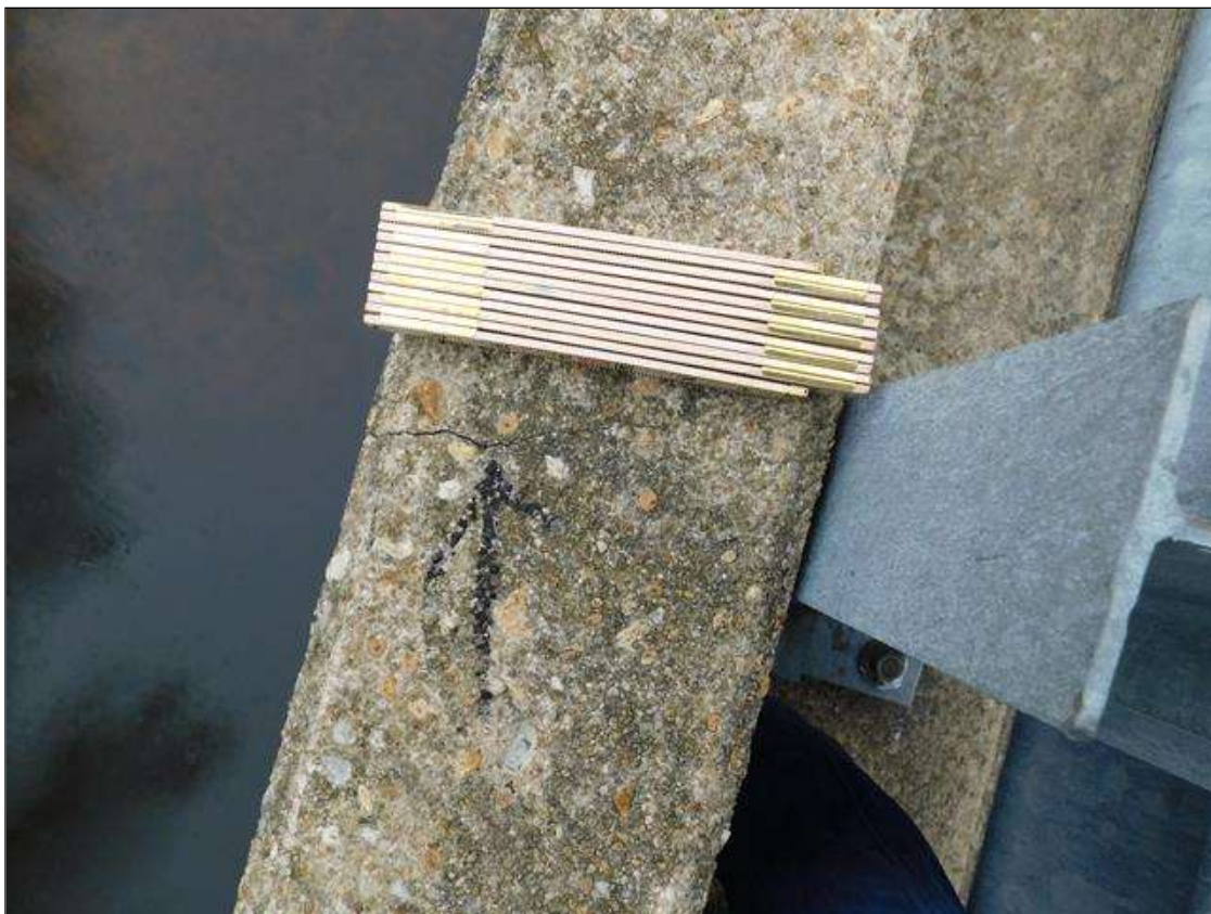
Span 2 Left Bridge Rail: (4) hairline vertical and transverse cracks on concrete rail and curb
