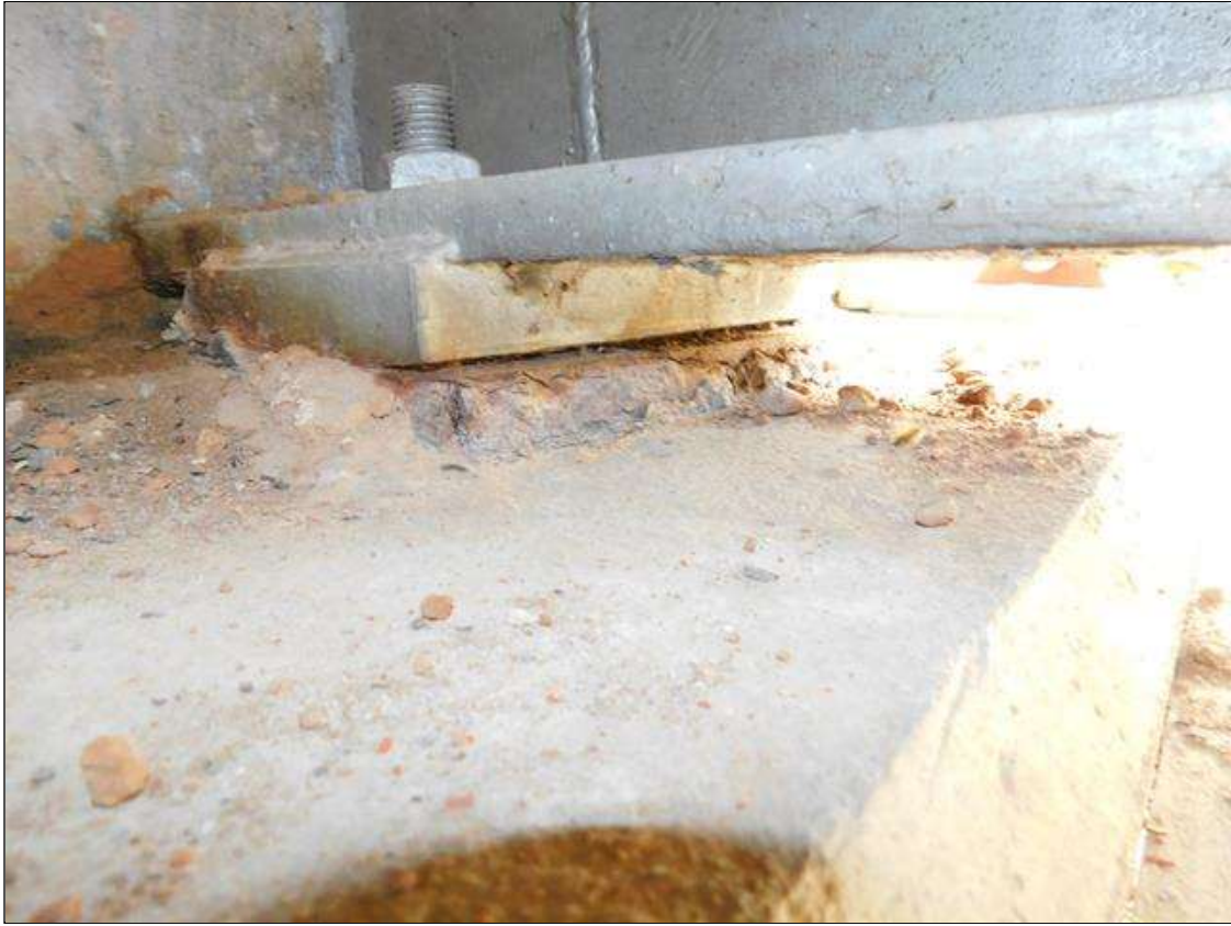
Span 1 Beam 1 Near Bearing: Peeling paint with rust
