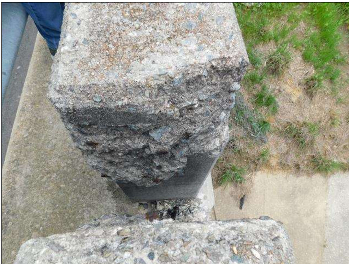
Span 4 Right Bridge Rail: 2" x 8" x 10" deep spall with exposed rebar on concrete Post 7 (Post 6 similar)
