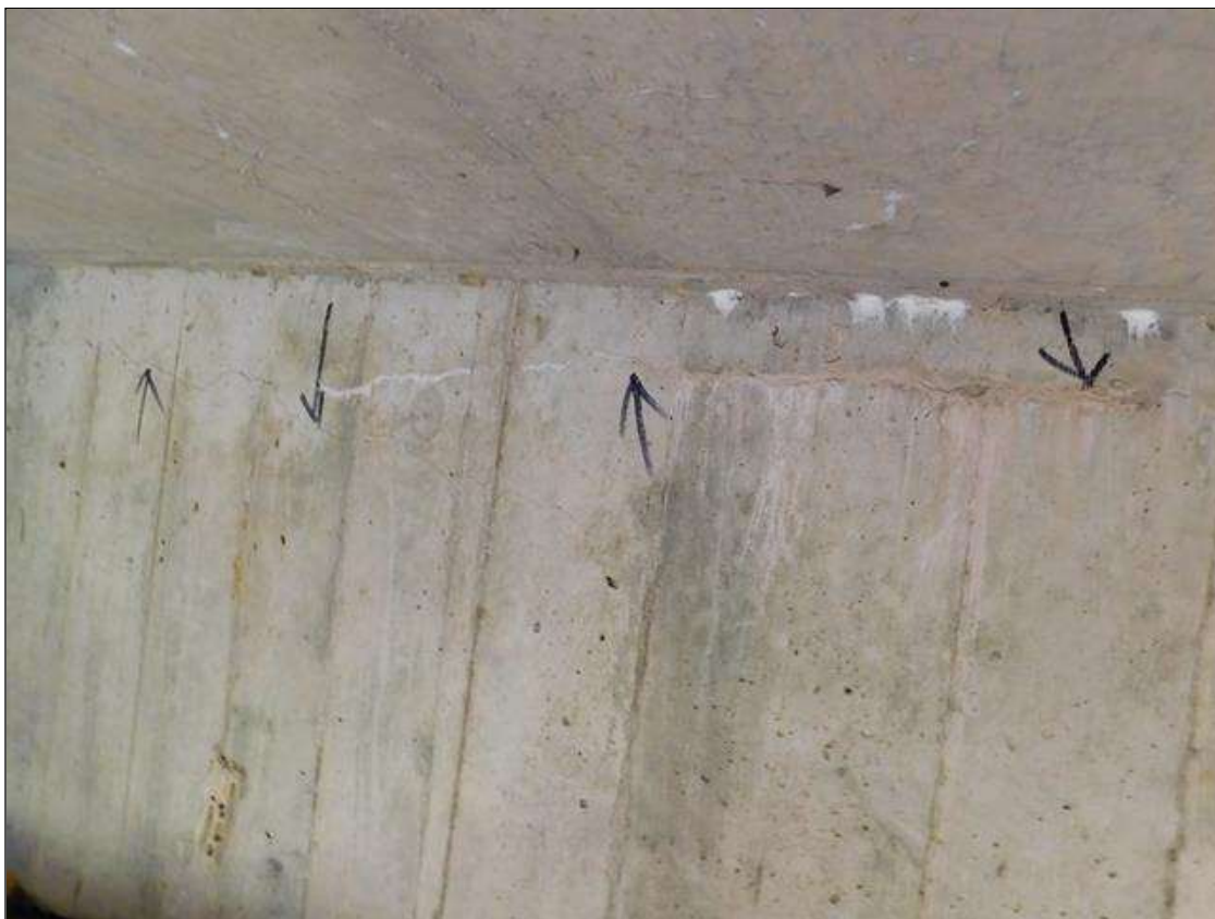
End Bent 2 Abutment/Backwall : 7' hairline horizontal crack with efflorescence in Bay 3
