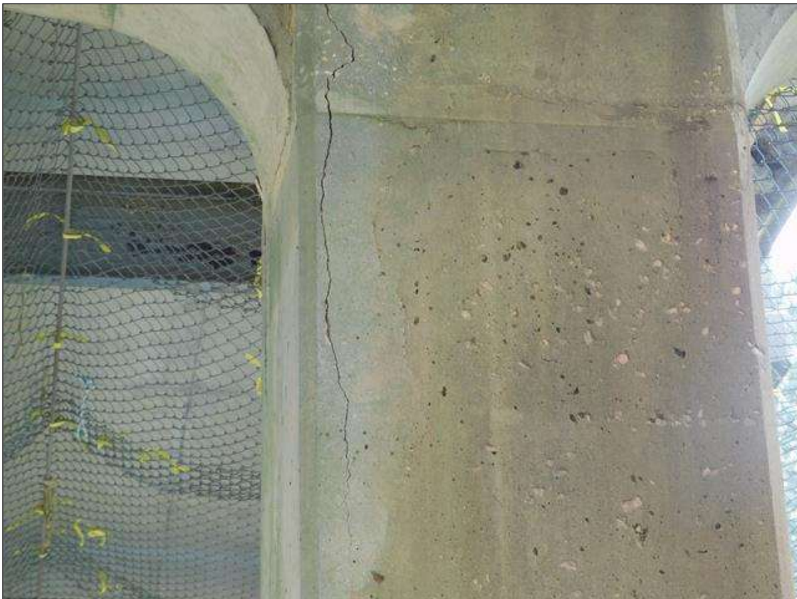
Bent 3 Pile 1: 3' up to 1/16" vertical crack on Span 4 face (East face similar)
