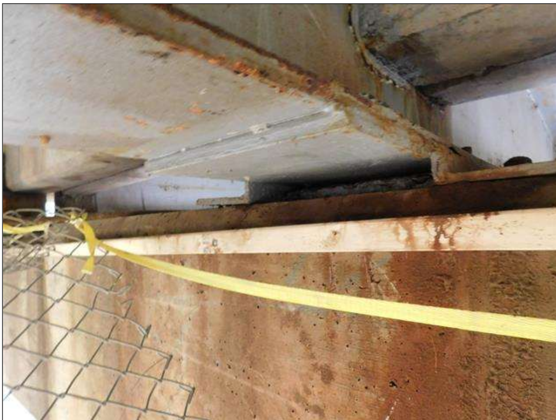
Span 1 Beam 2: Temporary Repair - 20" x 12" plate welded to bottom flange at Bent 1
