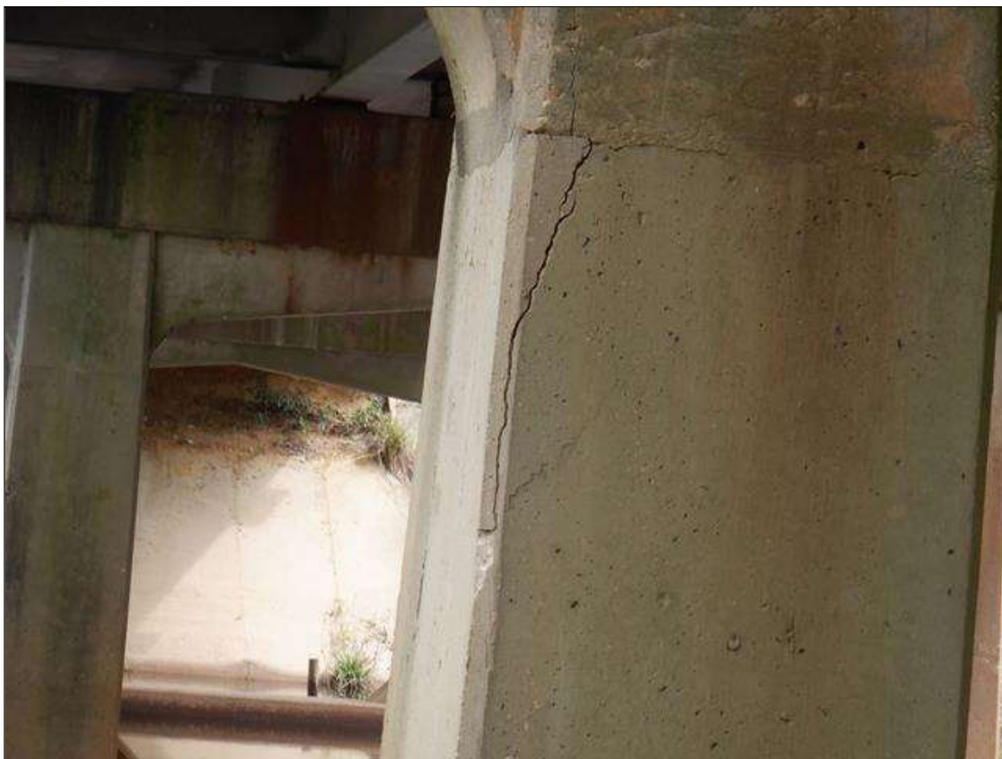
Bent 1 Pile 1: 42 INCHES X UP TO 1/4 INCHES VERTICAL CRACK WITH ADJACENT 4 FEET X UP TO 5 INCHES X 3 INCHES DELAMINATION ON SPAN 1 FACE
