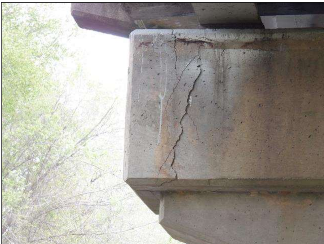
Bent 1 Cap 1: 12 INCHES X 24 INCHES AREA OF DELAMINATION WITH UP TO 1/8 INCHES VERTICAL AND DIAGONAL CRACKS ON SPAN 1 FACE AT WEST END
