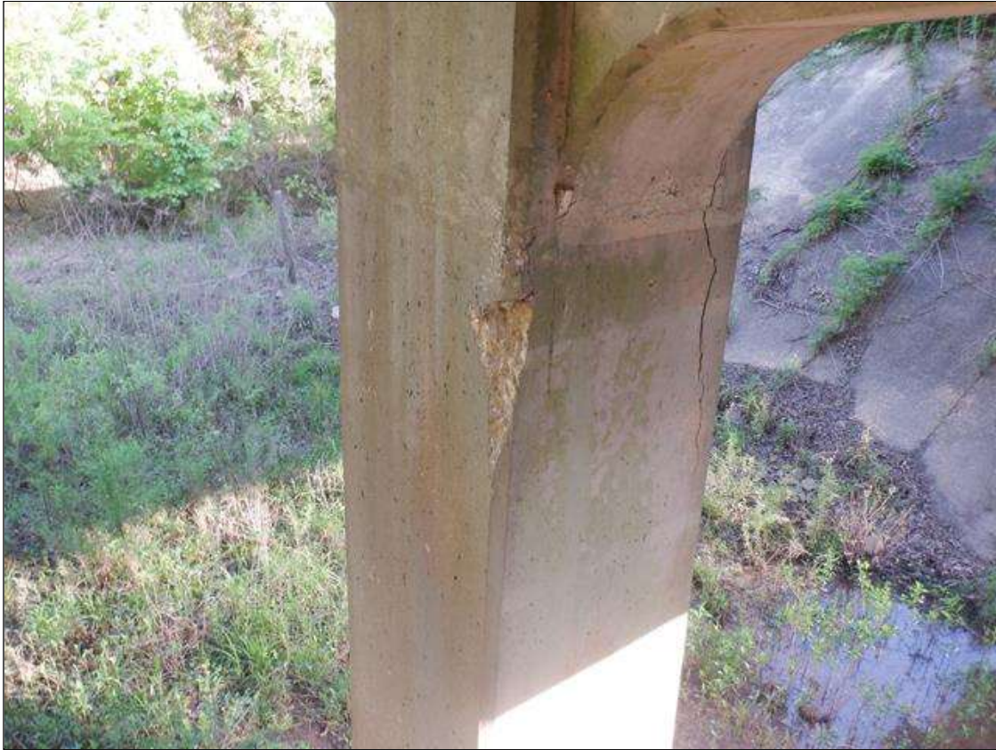
Bent 3 Pile 1: 14 INCHES X UP TO 6 INCHES X 2 INCHES SPALL WITH ADJACENT 1 FEET DIAMETER DELAMINATION ON SOUTHEAST CORNER, 2 FEET FROM BOTTOM OF CAP
