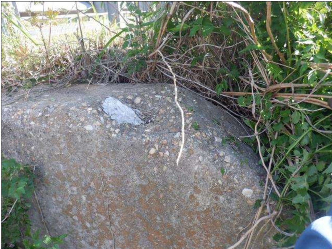
Wingwalls: 2 FEET X UP TO 1 FOOT X 2 INCHES SPALL IN TOP OF NORTHEAST WINGWALL.
