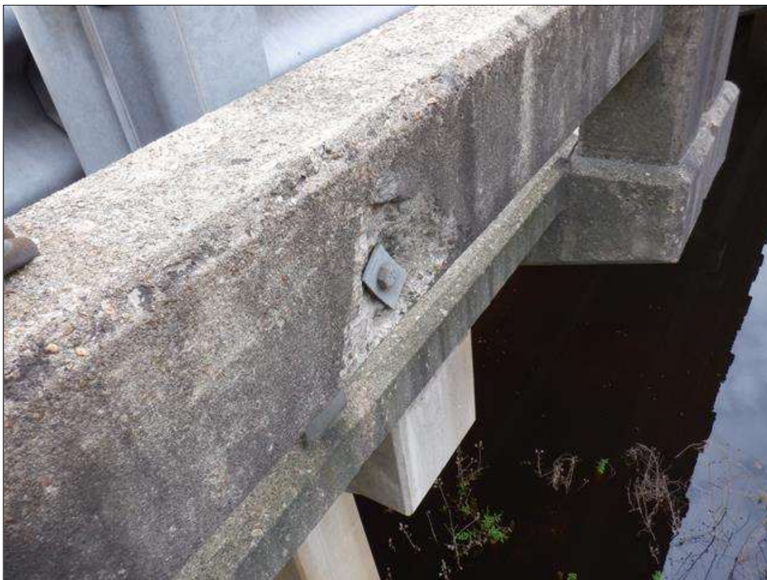
Span 4 Left Concrete Rail: (4) UP TO 10 INCHES X 9 INCHES X 1 INCHES DEEP SPALLS IN OUTSIDE FACE OF CONCRETE RAIL, AT RANDOM
