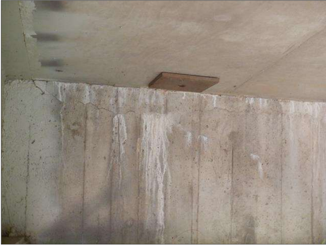
End Bent 2 Abutment: 7 FEET X UP TO 1/16 INCHES HORIZONTAL CRACK WITH EFFLORESCENCE IN BAY 3
