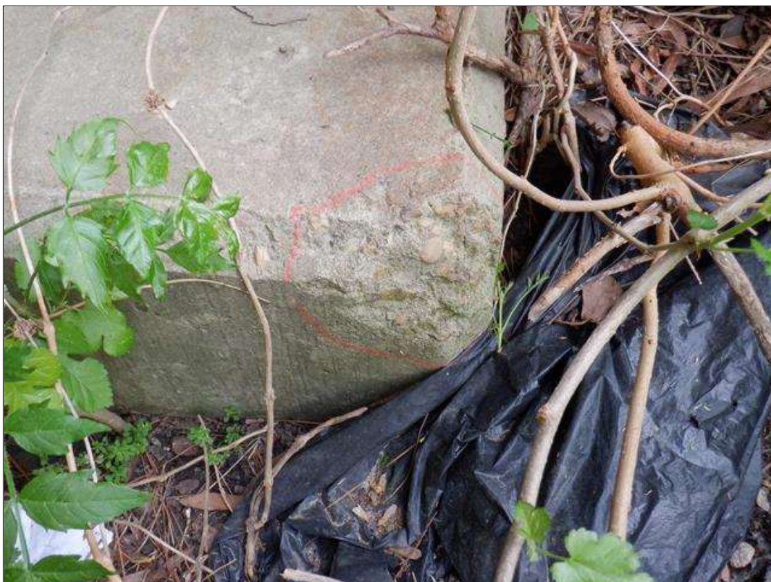
End Bent 1 Cap 1: 4 INCHES X 4 INCHES X 2 INCHES DEEP SPALL IN BRACE PILE CAP 1.
