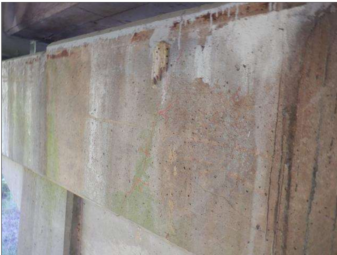
Bent 3 Cap 1: 12 FEET OF VERTICAL AND HORIZONTAL CRACKS UP TO 1/32 INCHES AT RANDOM THROUGHOUT
