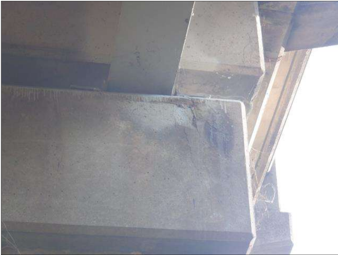
Bent 3 Cap 1: 4 INCHES X 6 INCHES X 1 INCHES DEEP SPALL WITH EXPOSED REBAR WITH ADJACENT UP TO 1/16 INCHES MAP CRACKING ON SPAN 3 FACE AT EAST END
