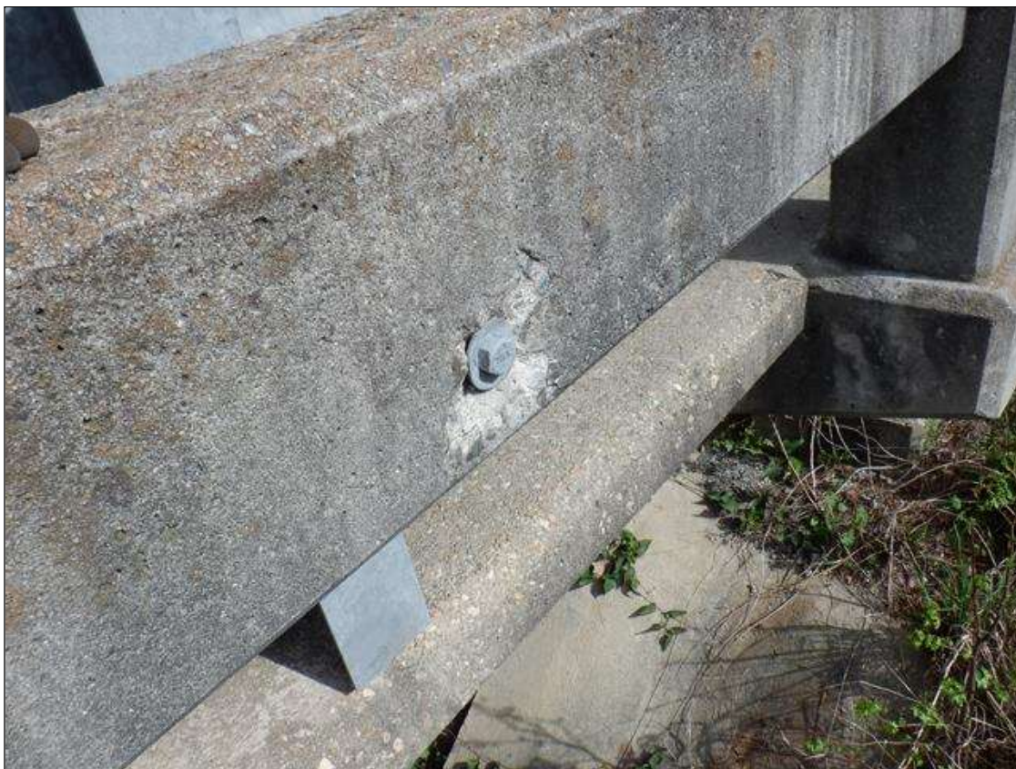
Span 4 Right Concrete Rail: 5 INCHES X 4 INCHES X 1/2 INCHES DEEP SPALL ON OUTSIDE FACE OF CONCRETE RAIL BETWEEN POSTS 7 & 8.
