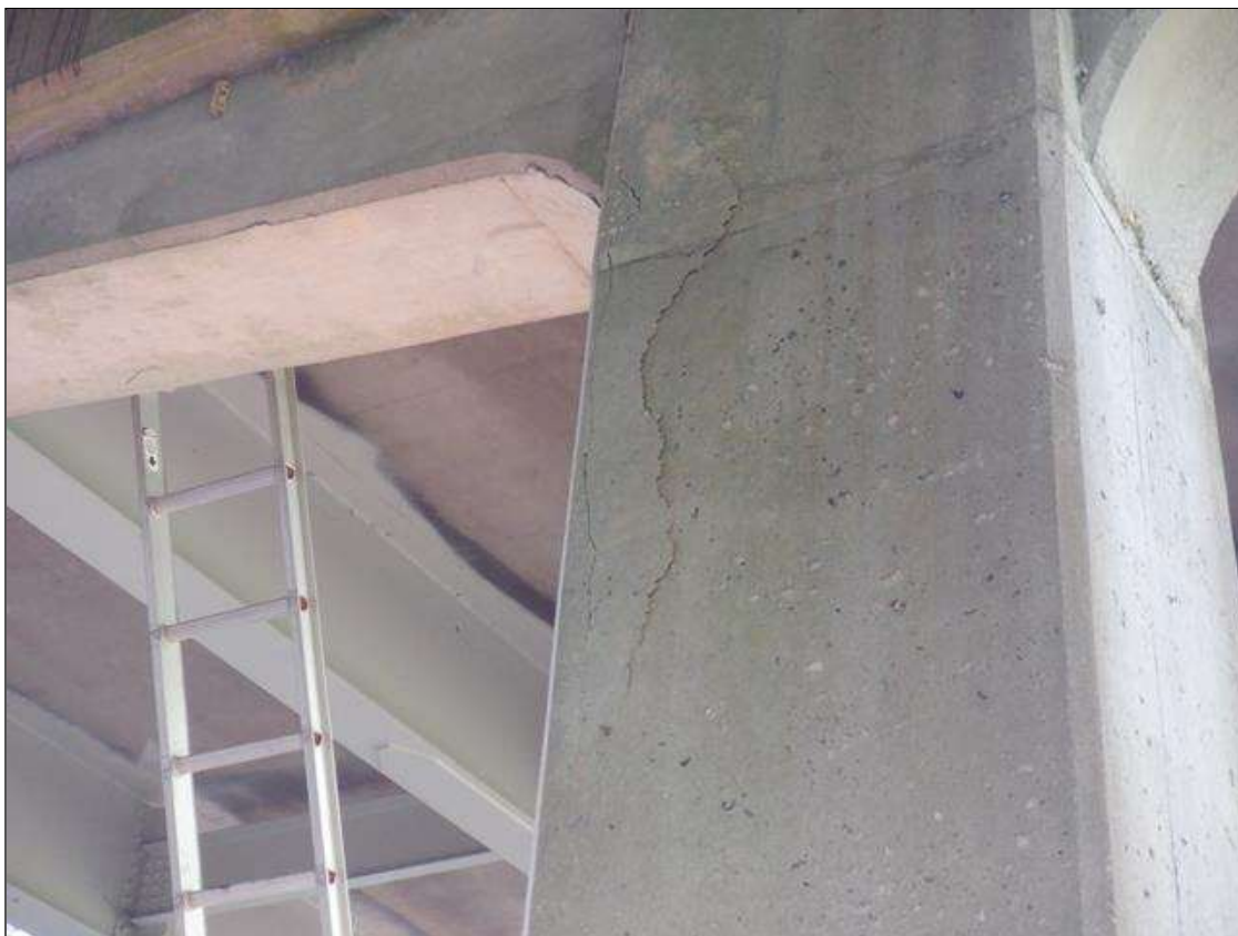
Bent 3 Pile 1: 6 FEET X UP TO 1 FEET X 8 INCHES DELAMINATION WITH UP TO 1/16 INCHES CRACKING AT NORTHEAST CORNER, 2 FEET BELOW CAP.
