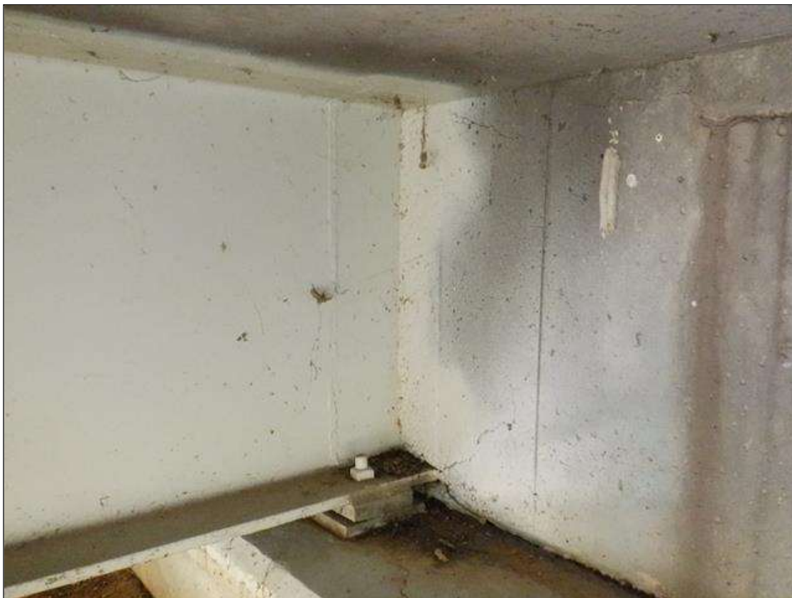
Span 1 Beam 3: 7 INCHES X 31 INCHES AREA OF REPLACED BEAM AT END BENT 1 (OTHER BEAMS AT END BENT 1 SIMILAR)
