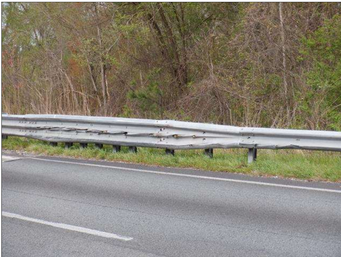
General Comments and Misc. Items: (PAR) 20 FEET OF IMPACT DAMAGE WITH 12- UP TO 10 INCHES X 1.5 INCHES GOUGES IN NORTHWEST GUARDRAIL, 15 FEET FROM END BENT 2.
