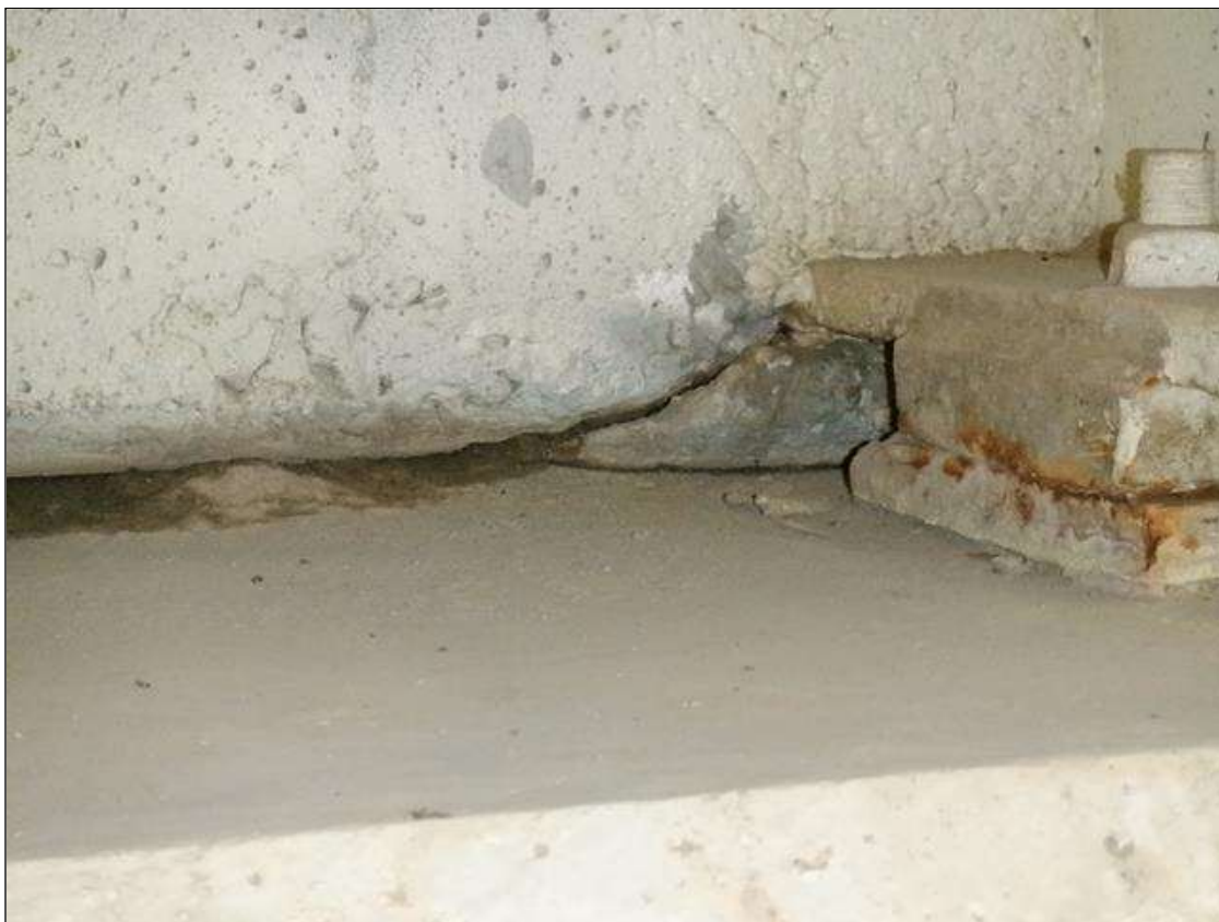
End Bent 1 Abutment: 8 INCHES X UP TO 1/4 INCHES DIAGONAL CRACK WITH ADJACENT 5 INCHES X UP TO 3 INCHES DELAMINATION ADJACENT TO BEAM 1. (ADJACENT TO ALL BEAMS SIMILAR)
