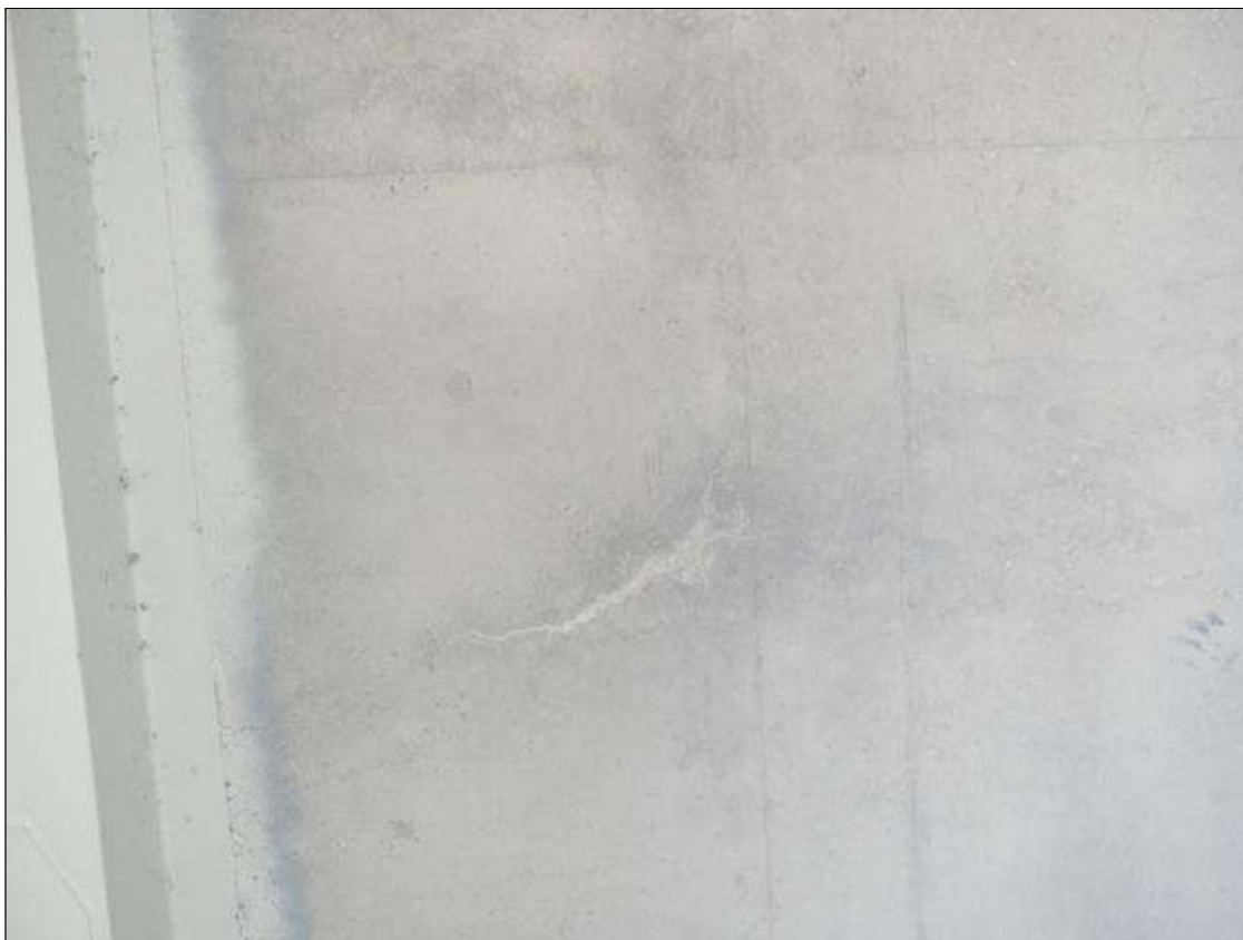
Span 3 Deck: 400 SQUARE FEET OF MAP CRACKING UP TO 1/32 INCHES, SOME WITH EFFLORESCENCE, AT RANDOM THROUGHOUT UNDERSIDE OF DECK (PHOTO TAKEN IN BAY 3)
