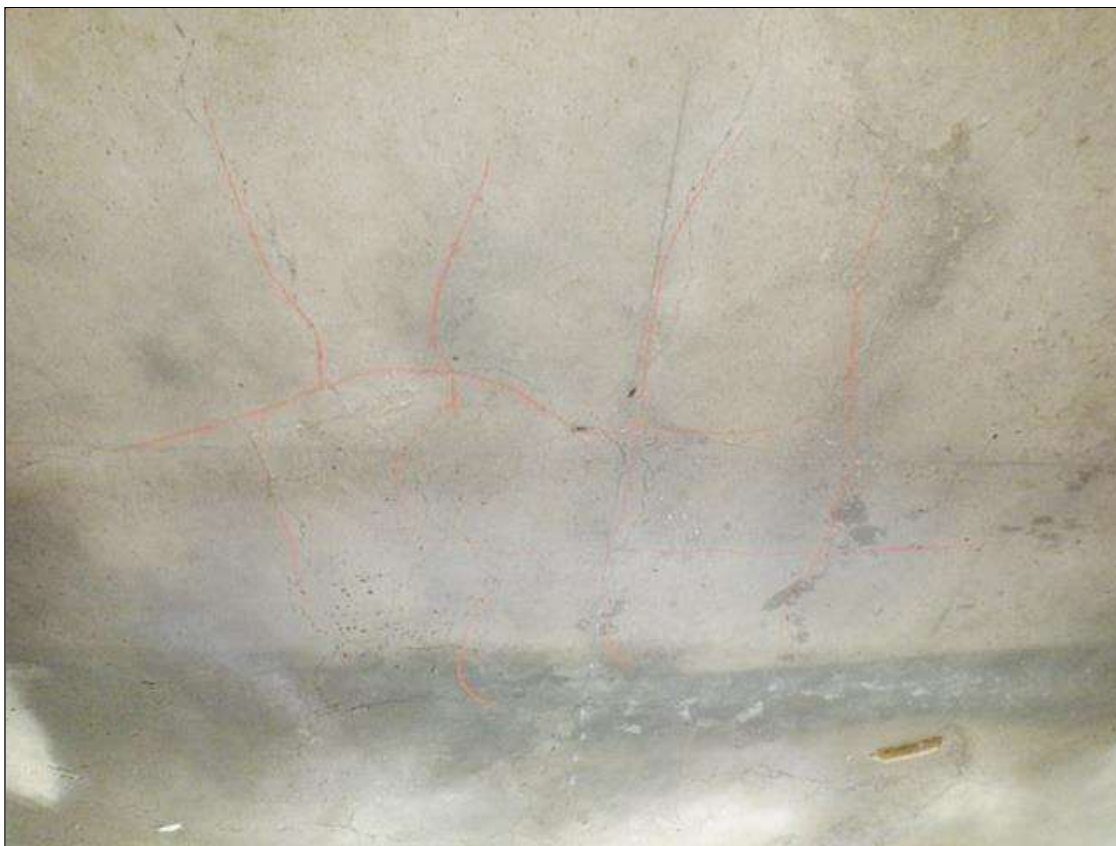
Span 1 Deck: 400 SQUARE FEET OF MAP CRACKING UP TO 1/32 INCHES AT RANDOM THROUGHOUT UNDERSIDE OF DECK (PHOTO TAKEN IN BAY 2)
