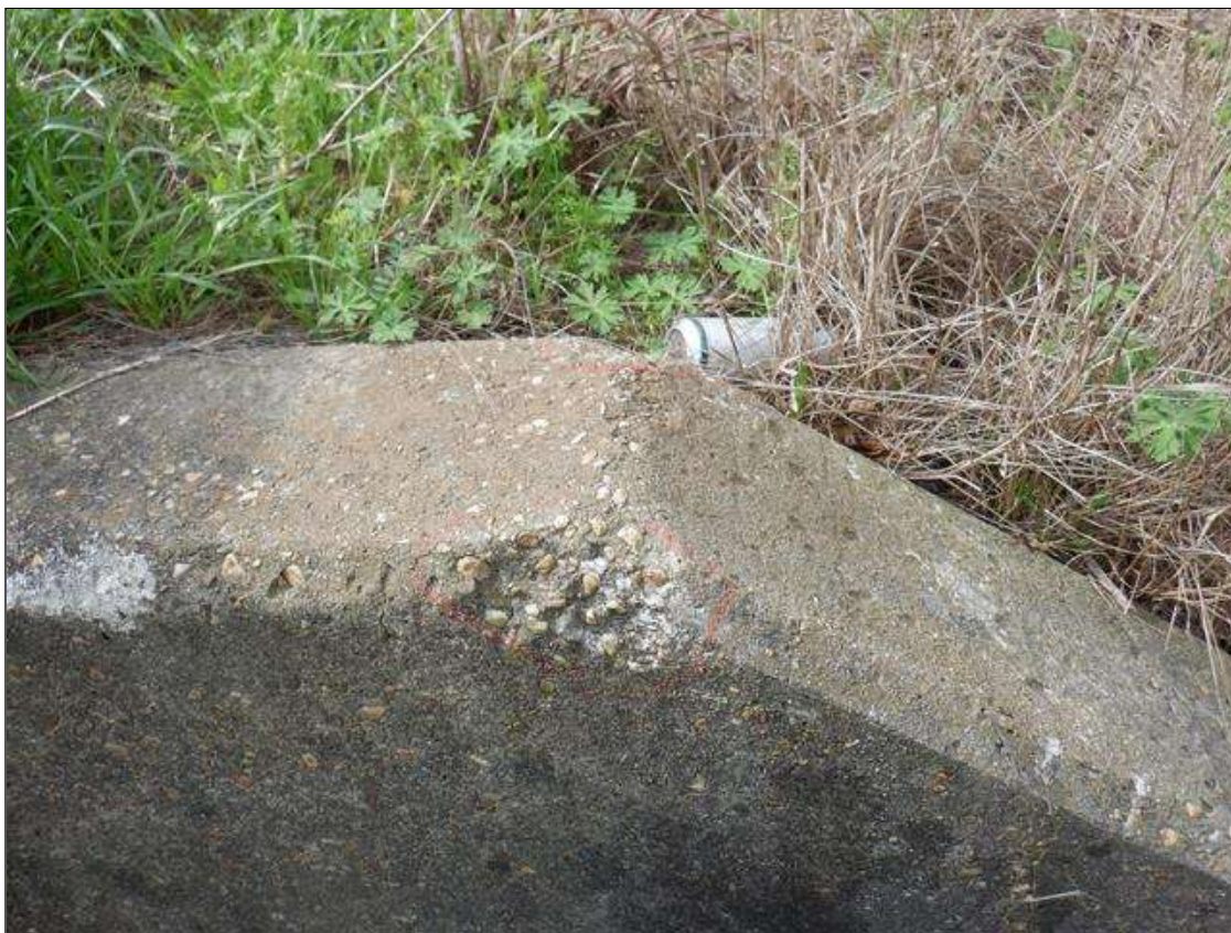
Wingwalls: 2- UP TO 6 INCHES X 3 INCHES X 1 INCHES SPALLS IN TO OF SOUTHWEST WINGWALL
