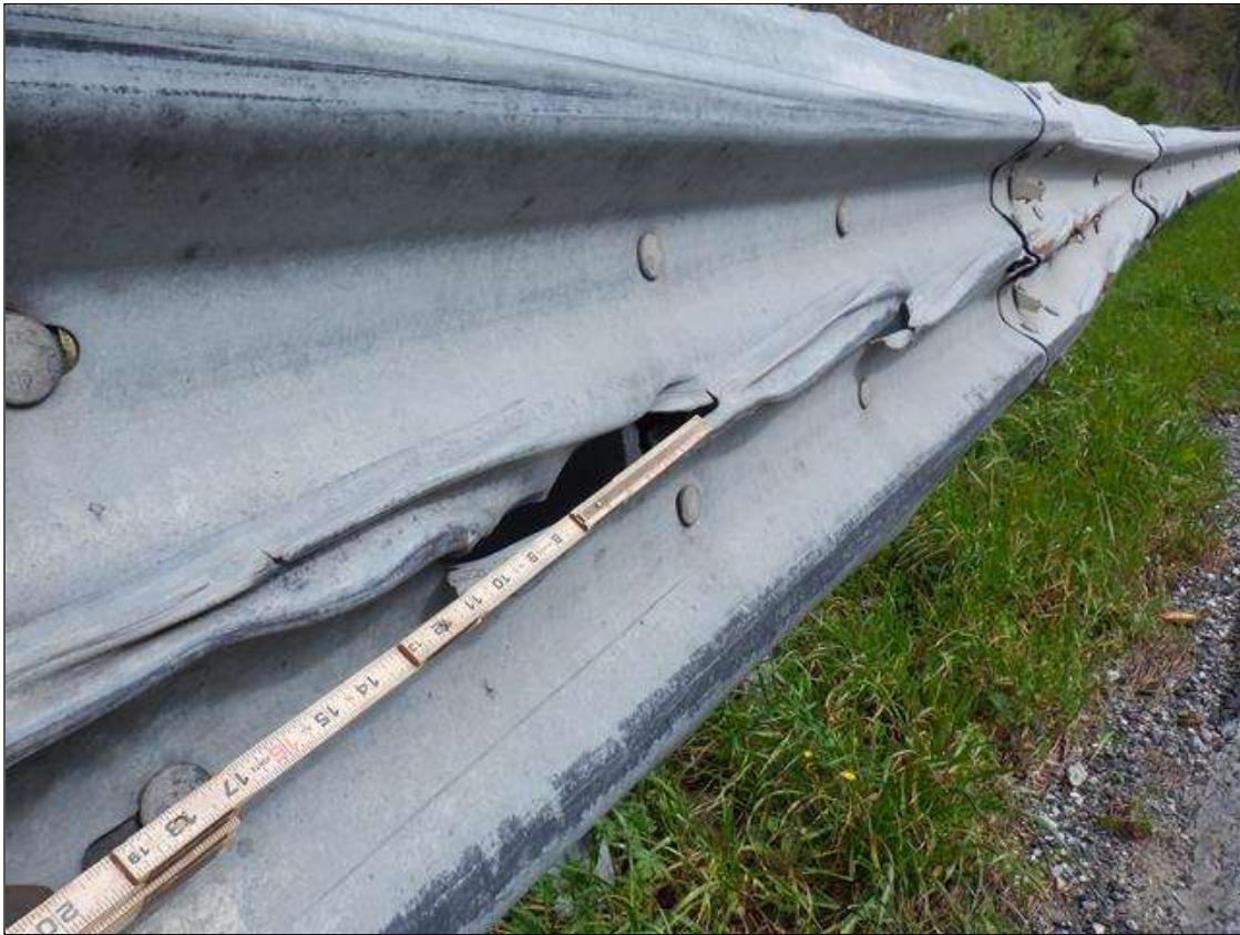
General Comments and Misc. Items: (PAR) 20 FEET OF IMPACT DAMAGE WITH 12- UP TO 10 INCHES X 1.5 INCHES GOUGES IN NORTHWEST GUARDRAIL, 15 FEET FROM END BENT 2.
