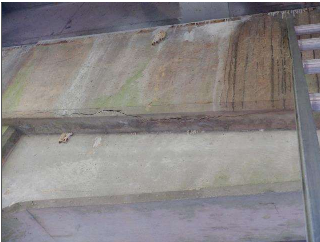
Bent 3 Cap 1: 6 FEET X UP TO 1/8 INCHES HORIZONTAL CRACK ON SOUTH BOTTOM FACE UNDER BEAM 2
