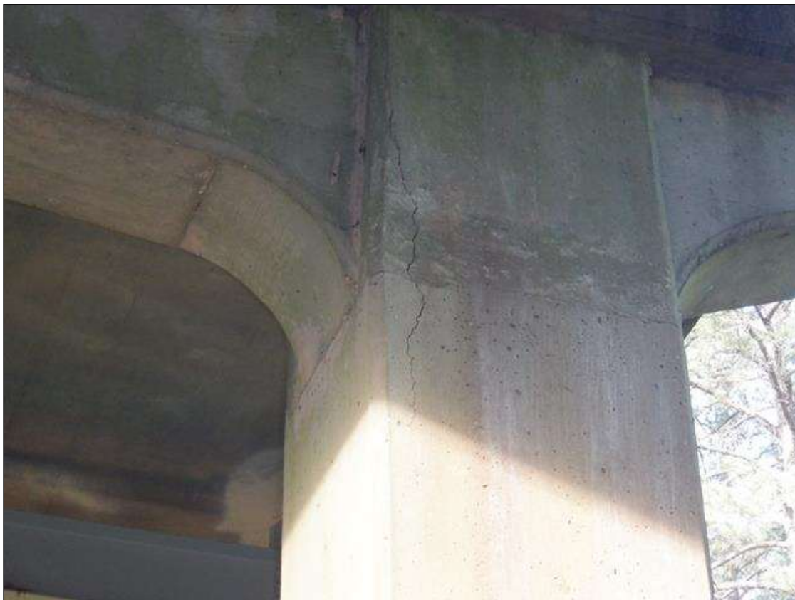
Bent 1 Pile 1: 6 FEET X UP TO 1/8 INCHES VERTICAL CRACK IN NORTHEAST CORNER, 1 FOOT FROM BOTTOM OF CAP.
