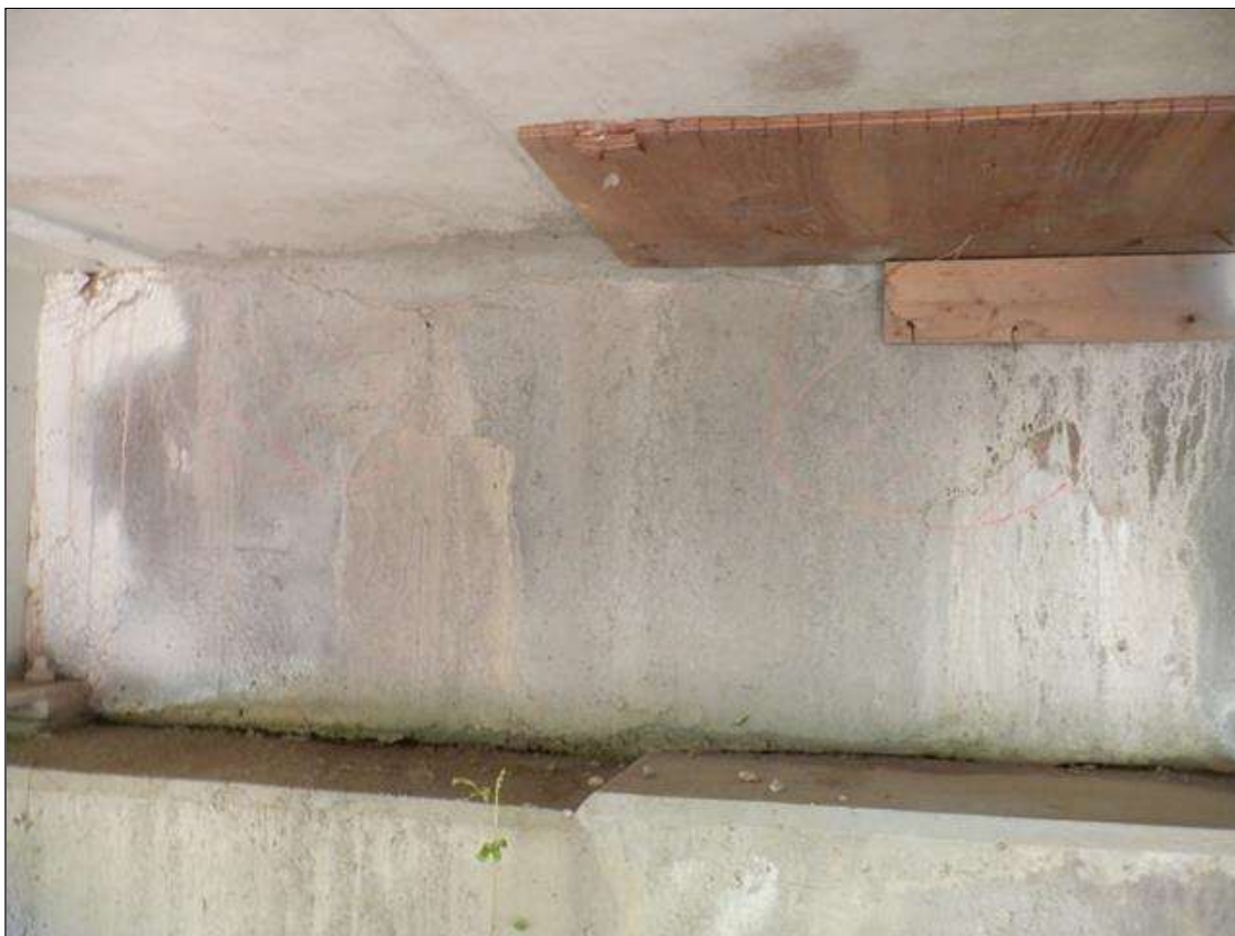
End Bent 2 Abutment: (2) UP TO 24 INCHES X 12 INCHES AREAS OF DELAMINATION IN BAY 1
