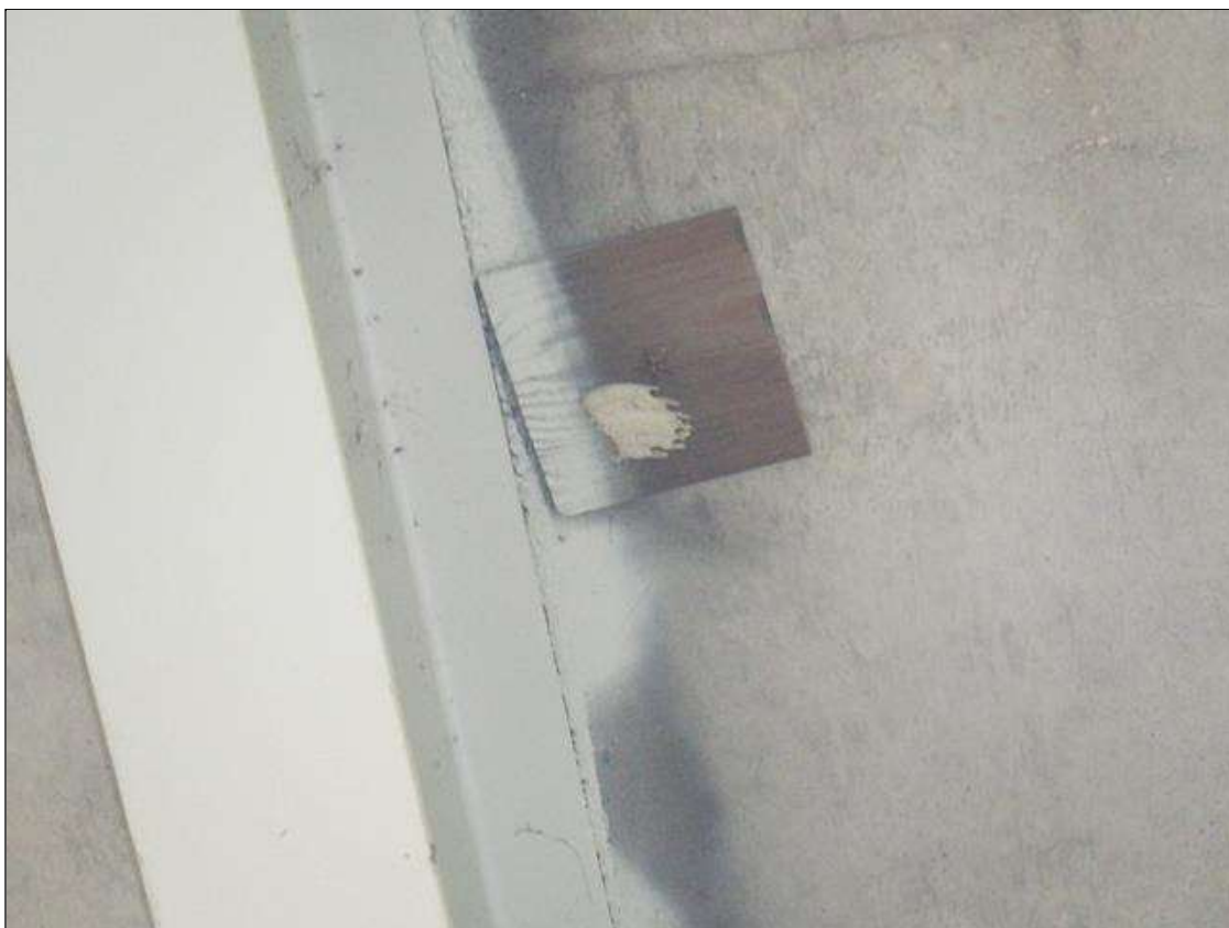
Span 3 Deck: 1 FEET X 1 FEET TIMBER PATCH IN BAY 2, 8 FEET FROM BENT 2, ADJACCENT TO BEAM 3.
