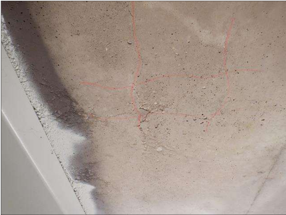
Span 4 Deck: 400 SQUARE FEET OF MAP CRACKING UP TO 1/32 INCHES AT RANDOM THROUGHOUT UNDERSIDE OF DECK
