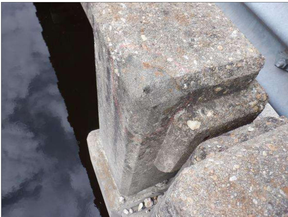
Span 2 Right Concrete Rail: 4 INCHES X 3 INCHES X UP TO 3 INCHES SOUND PATCHED AREA ON TOP OF POST
