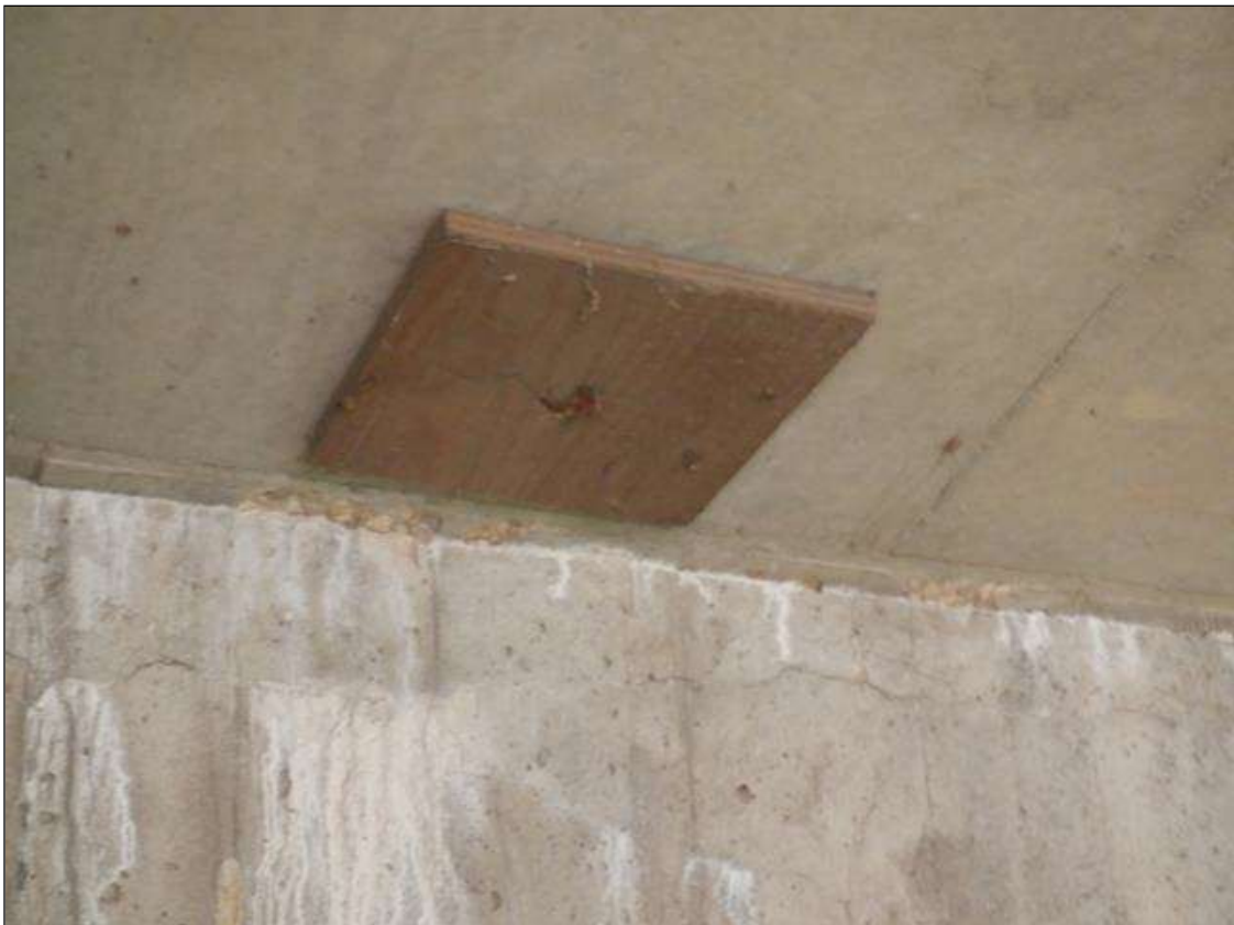
Span 4 Deck: 1 FEET X 1 FEET TIMBER PATCH IN BAY 3 AT END BENT 2.
