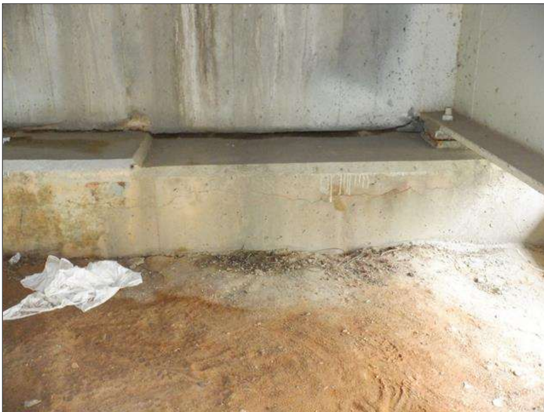
End Bent 1 Cap 1: 5 FEET UP TO 1/32 INCHES HORIZONTAL CRACK WITH RUST STAINING UNDER BAY 1
