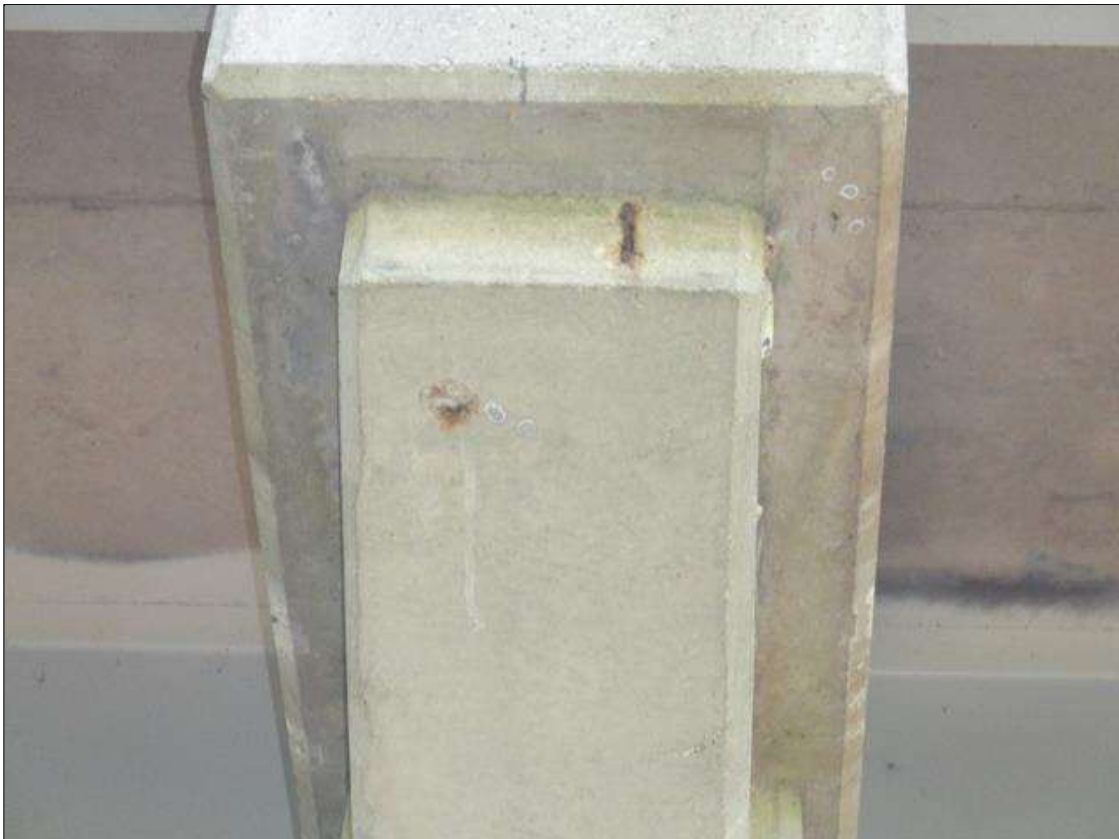
Bent 3 Pile 1: (2) UP TO 3 INCHES X 6 INCHES X 1 INCHES DEEP SPALLS WITH EXPOSED REBAR ON WEST AND BOTTOM FACE OF CORBEL.
