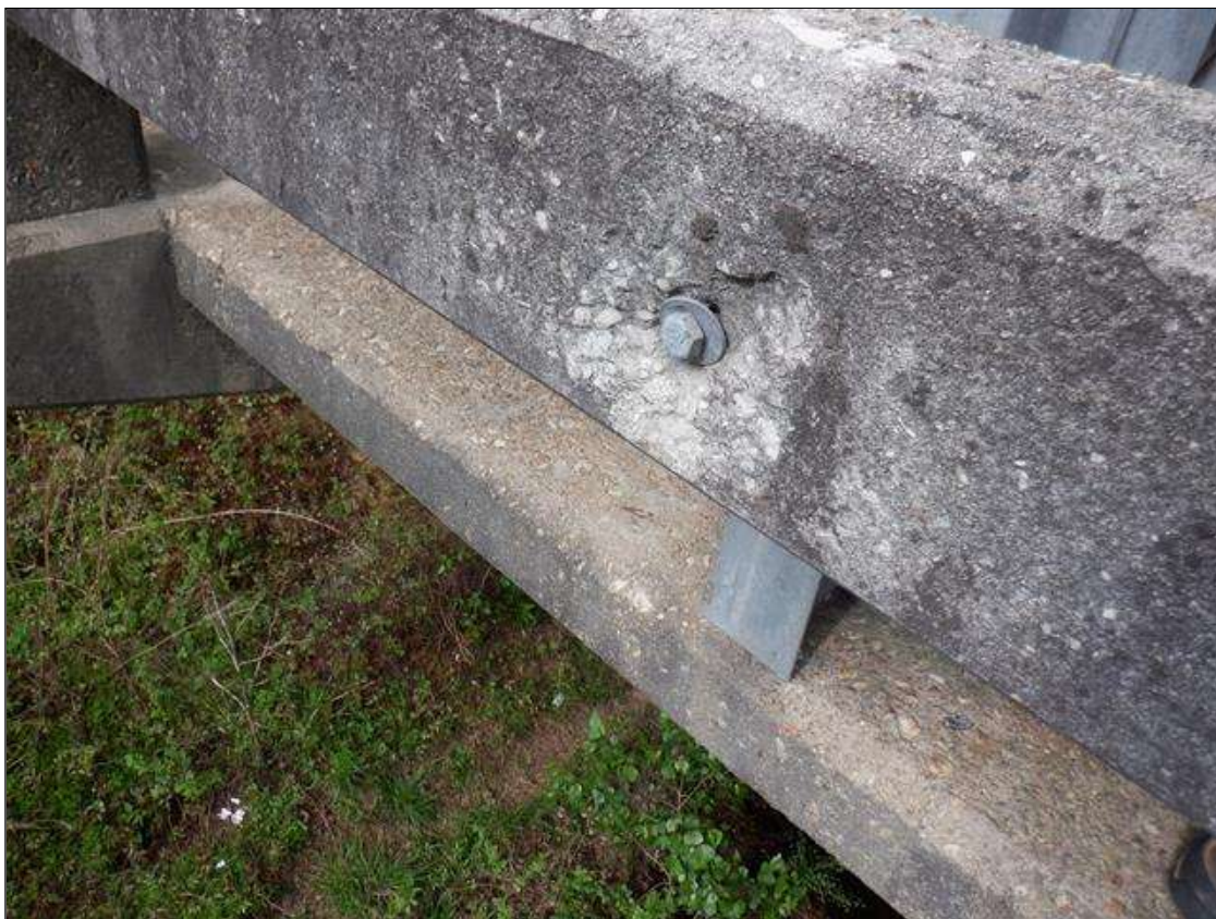
Span 1 Right Concrete Rail: 2- UP TO 7 INCHES X 6 INCHES X 1 INCHES SPALLS IN OUTSIDE FACE OF RAIL NEAR BENT 1
