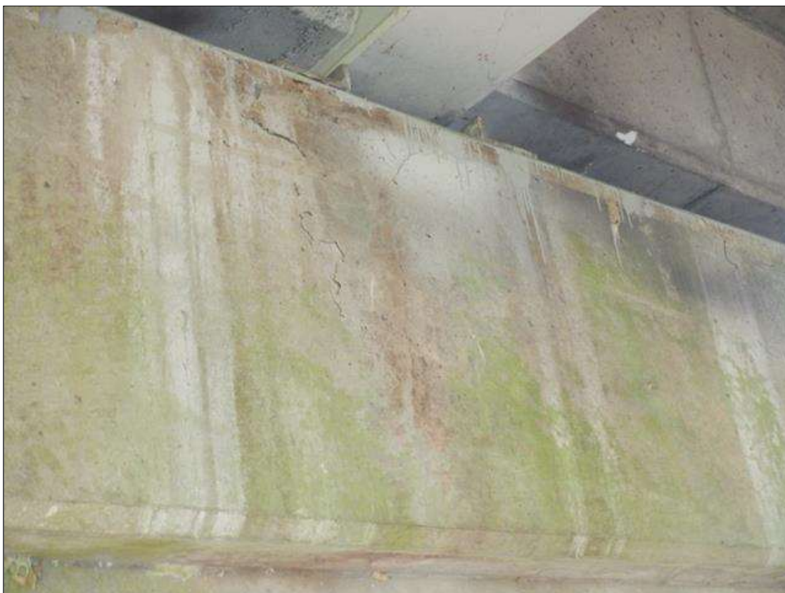
Bent 3 Cap 1: 3- UP TO 2 FEET X 20 INCHES DELAMINATIONS WITH UP TO 1/32 INCHES MAP CRACKING AT RANDOM THROUGHOUT SOUTH FACE (PHOTO TAKEN UNDER BEAM 2)
