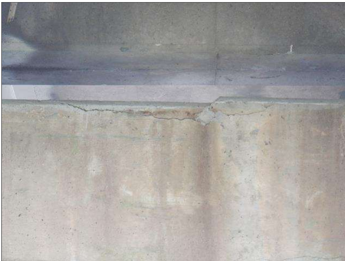
Bent 1 Cap 1: 3 FEET X UP TO 1/8 INCHES HORIZONTAL CRACK ON SPAN 1 FACE UNDER BAY 1
