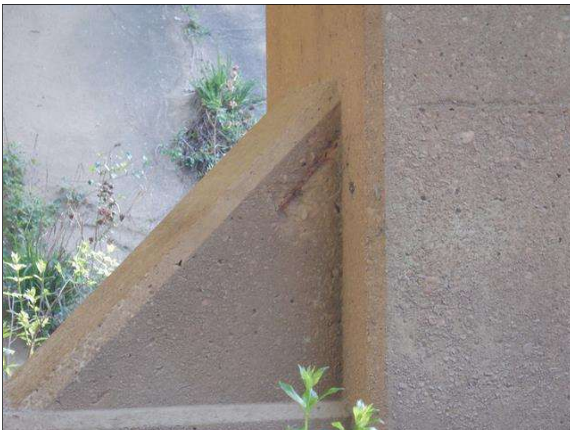
Bent 3 Pile 2: 8 INCHES X 4 INCHES X UP TO 1/2 INCHES SPALL WITH EXPOSED REINFORCING ON SPAN 3 FACE OF CORBEL UNDER STRUT.
