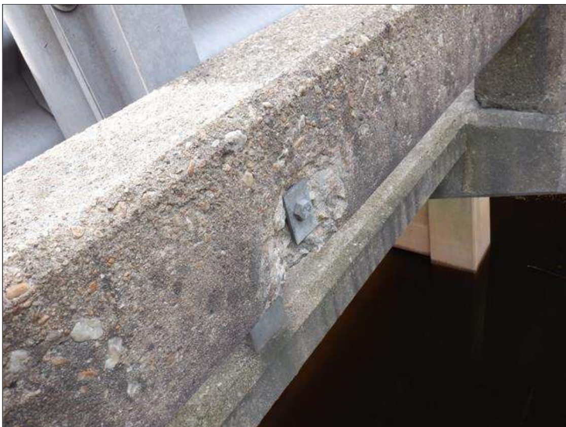
Span 2 Left Concrete Rail: (4) UP TO 9 INCHES X 6 INCHES X 1 INCHES DEEP SPALLS IN OUTSIDE FACE OF CONCRETE RAIL, AT RANDOM
