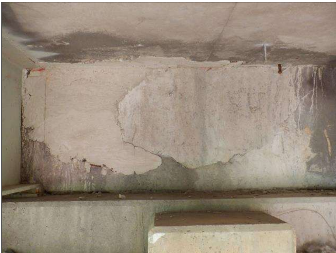
End Bent 2 Abutment: 8 FEET X 2 FEET AREA OF DELAMINATED PATCH IN BAY 2
