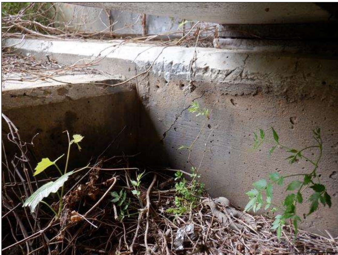
End Bent 1 Cap 1: 16 INCHES UP TO 1/16 INCHES DIAGONAL CRACK UNDER BEAM 4 (BELOW BEAM 1 SIMILAR)
