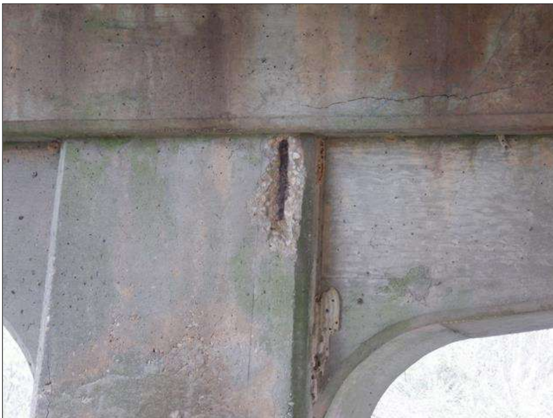
Bent 1 Pile 1: (PAR) 12 INCHES X 5 INCHES X 1 INCHES SPALL WITH EXPOSED REBAR ON SOUTH FACE AT BOTTOM OF CAP
