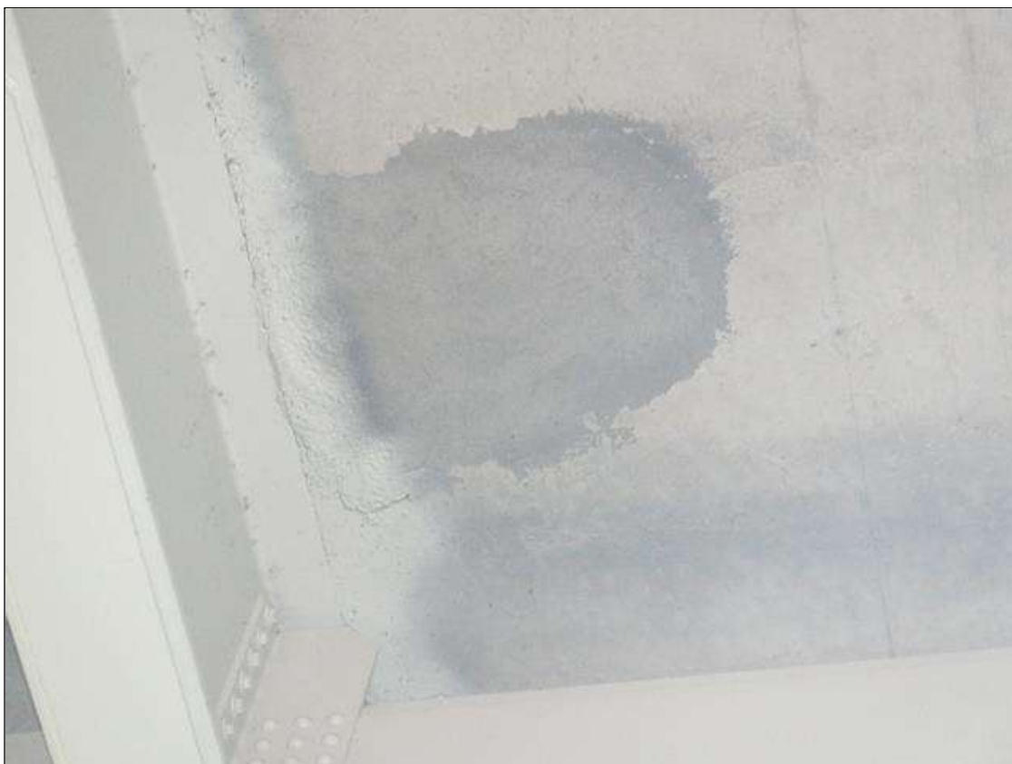
Span 3 Deck: 2.5 FEET X 2.5 FEET SOUND PATCH IN BAY 3, 16 FEET FROM BENT 2.
