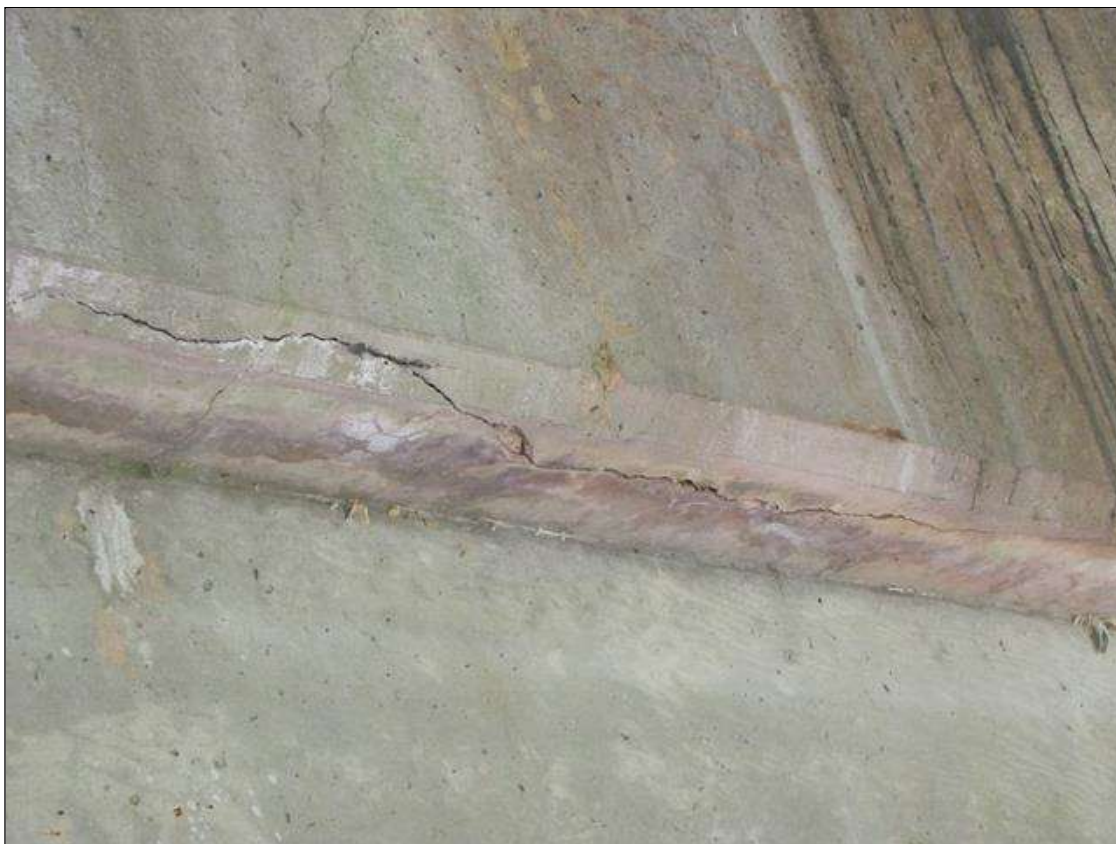
Bent 3 Cap 1: 4' up to 1/16" horizontal crack on Span 3 BOTTOM face UNDER BEAM 2
