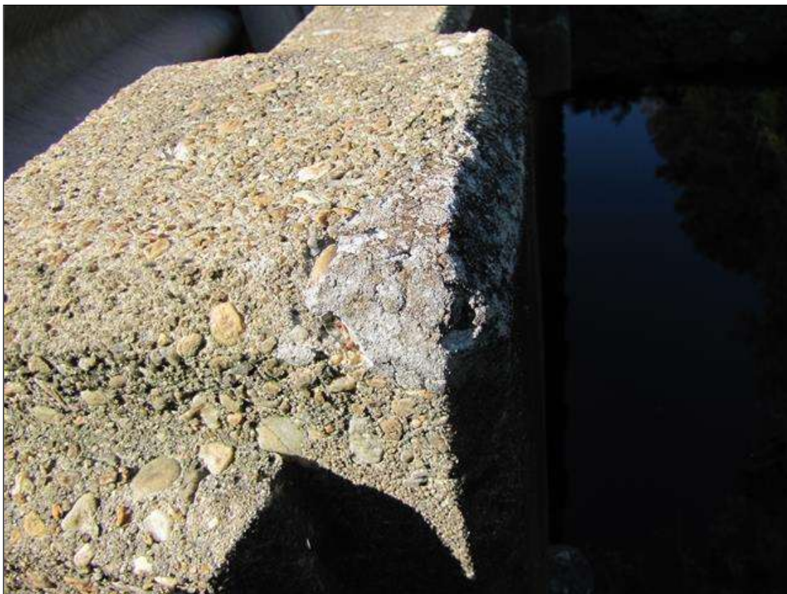
Span 3 Left Bridge Rail: 5" x 2" area of sound patch on top of concrete Post 3
