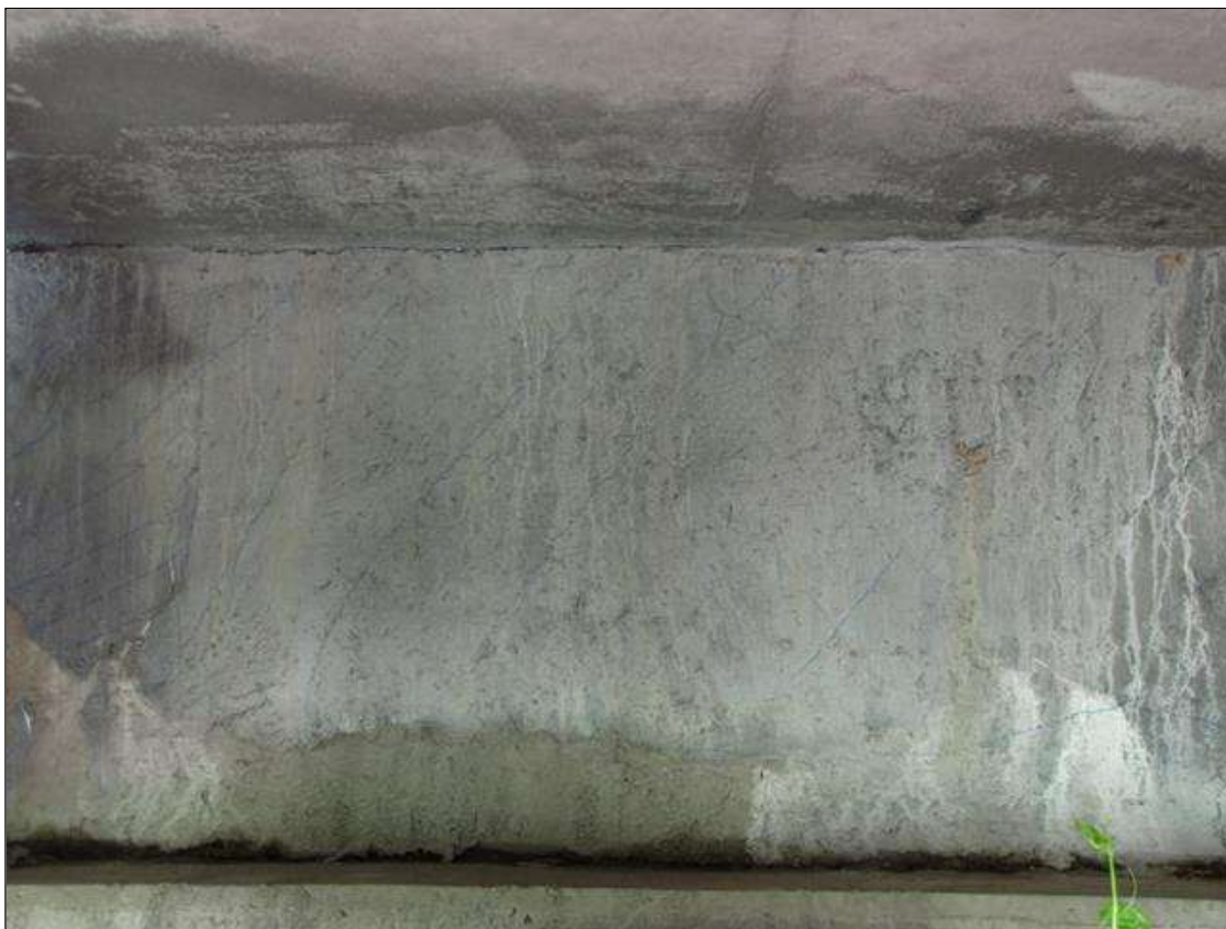
End Bent 2 Abutment/Backwall : 8' x 2' area of delaminated patch in Bay 2
