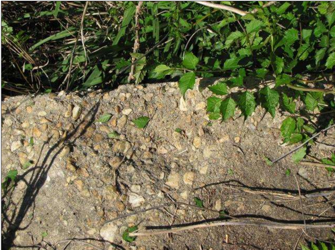
Wingwalls: UP TO 24" x 12" x 2" SPALL ON TOP OF NORTHEAST WINGWALL
