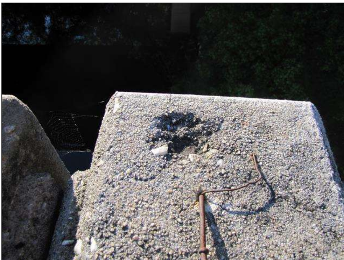
Span 1 Right Bridge Rail: 3" x 2" x 1/2" SPALL TOP OF POST 8
