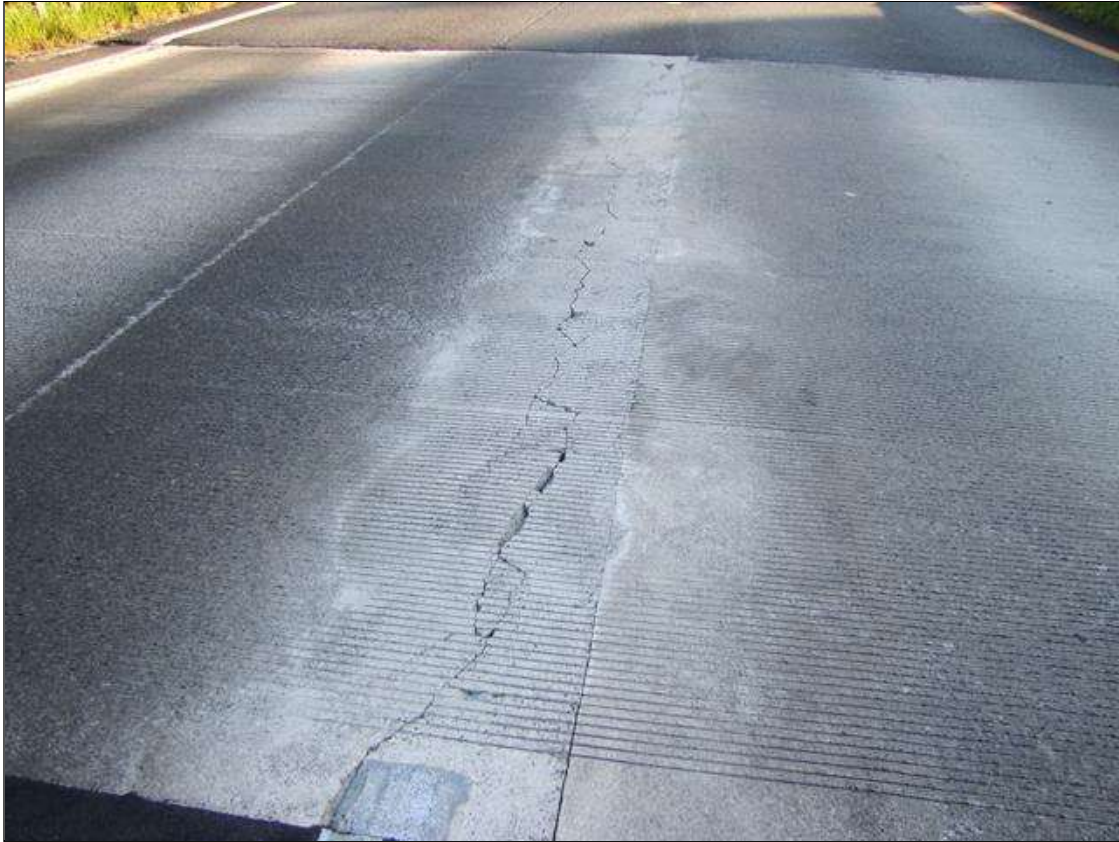
Approach 2: 25' X UP TO 1/8" LONGITUDINAL CRACK AT CENTERLINE OF ROADWAY
