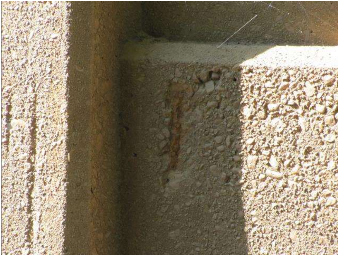
Bent 2 Pile 2: 2" x 6" x 1/2" deep spall with exposed rebar on Span 3 face of strut
