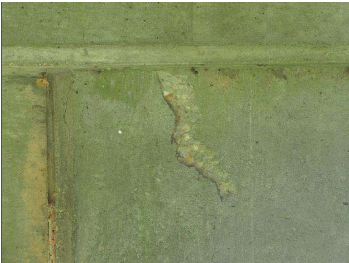
Bent 1 Pile 2: 8" X 2" X 1/4" SPALL AT BOTTOM OF CAP WITH ADJACENT 18" up to 1/16" vertical crack on Span 1 face
