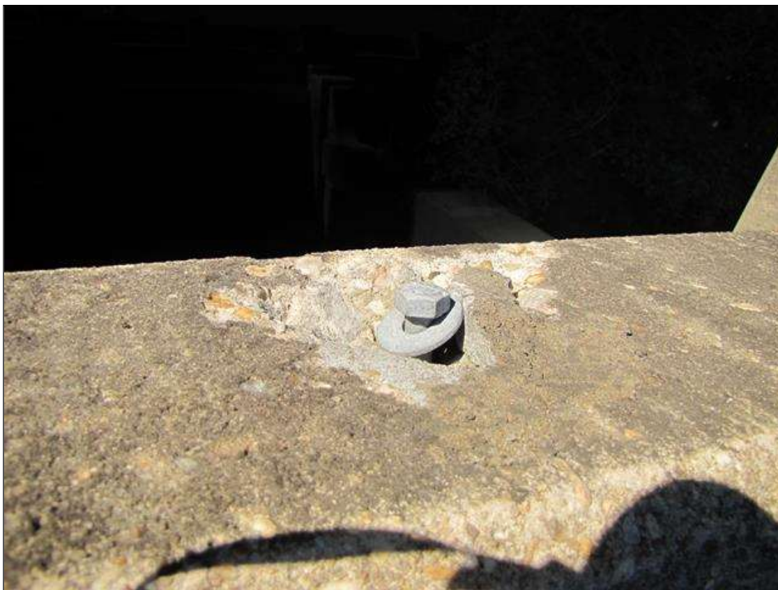
Span 2 Right Bridge Rail: 7" x 5" x 1" deep spall on outside face of concrete rail 10' FROM BENT 1
