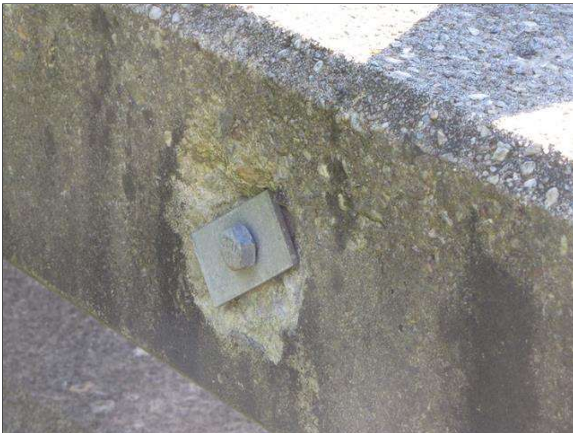
Span 1 Left Bridge Rail: (3) up to 10" x 6" x 1" deep spall on outside face of concrete rail (PHOTO TAKEN NEAR END BENT 1)
