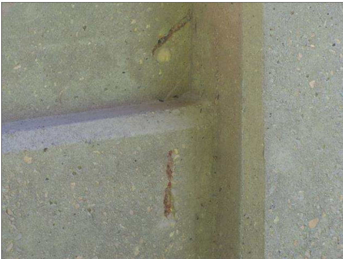
Bent 1 Pile 2: (2) up to 3" x 2" x 1/2" deep spall with exposed rebar on corbel and strut on Span 1 face
