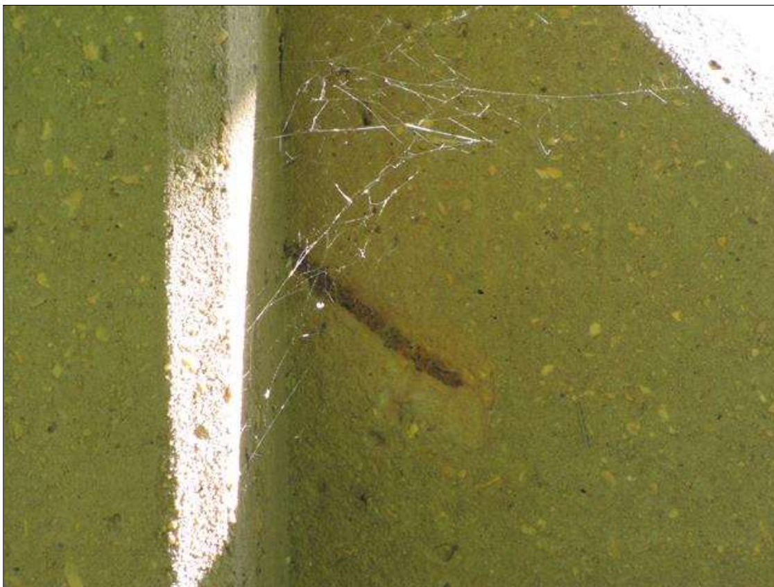
Bent 1 Pile 1: 2" x 6" x 1/2" deep spall with exposed rebar on Span 1 face of strut
