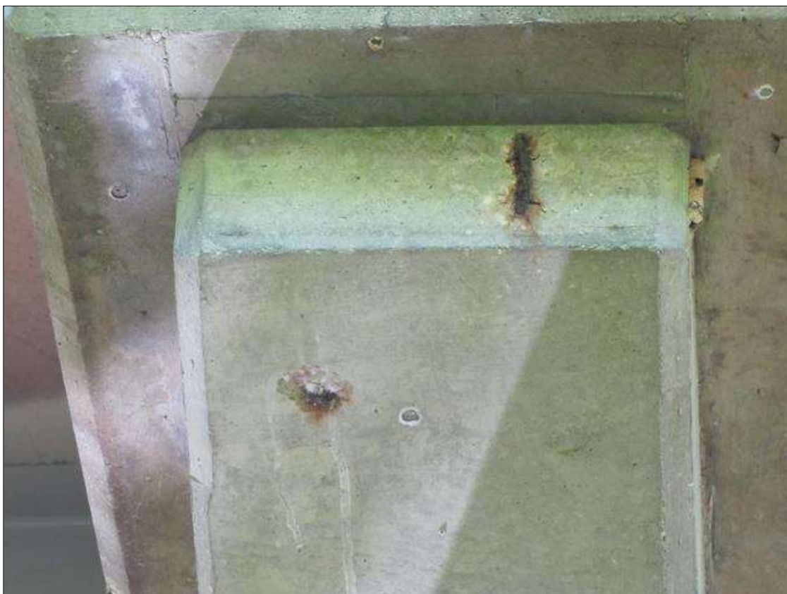
Bent 3 Pile 1: (2) up to 3" x 6" x 1" deep spall with exposed rebar on West face of corbel
