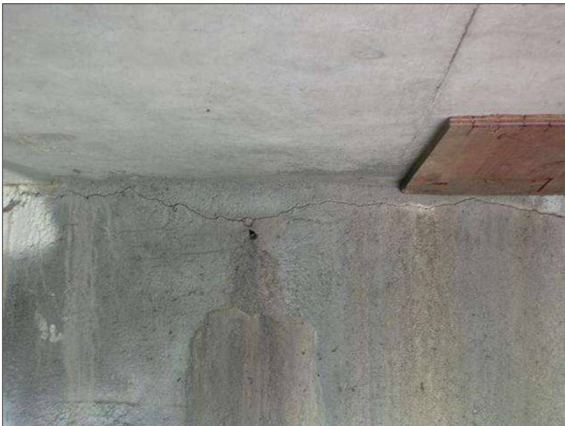
End Bent 2 Abutment/Backwall : 6' x up to 1/64" horizontal crack with efflorescence in Bay 1
