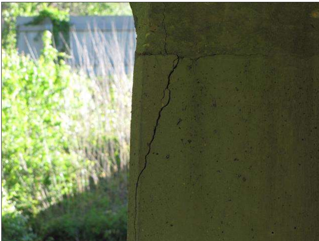
Bent 1 Pile 1: 30" up to 1/8" vertical crack on Span 1 face
