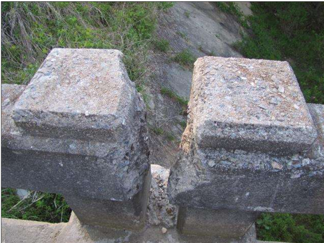
Span 4 Right Bridge Rail: 2" x 8" x 10" deep spall with exposed rebar on concrete Post 7 (Post 6 similar)
