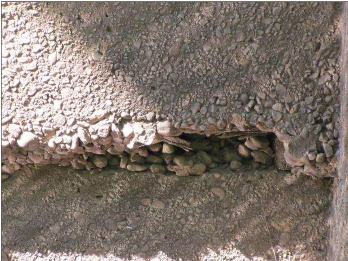
Bent 2 Pile 1: 10" x 2" x 2" deep spall on Span 3 face of strut
