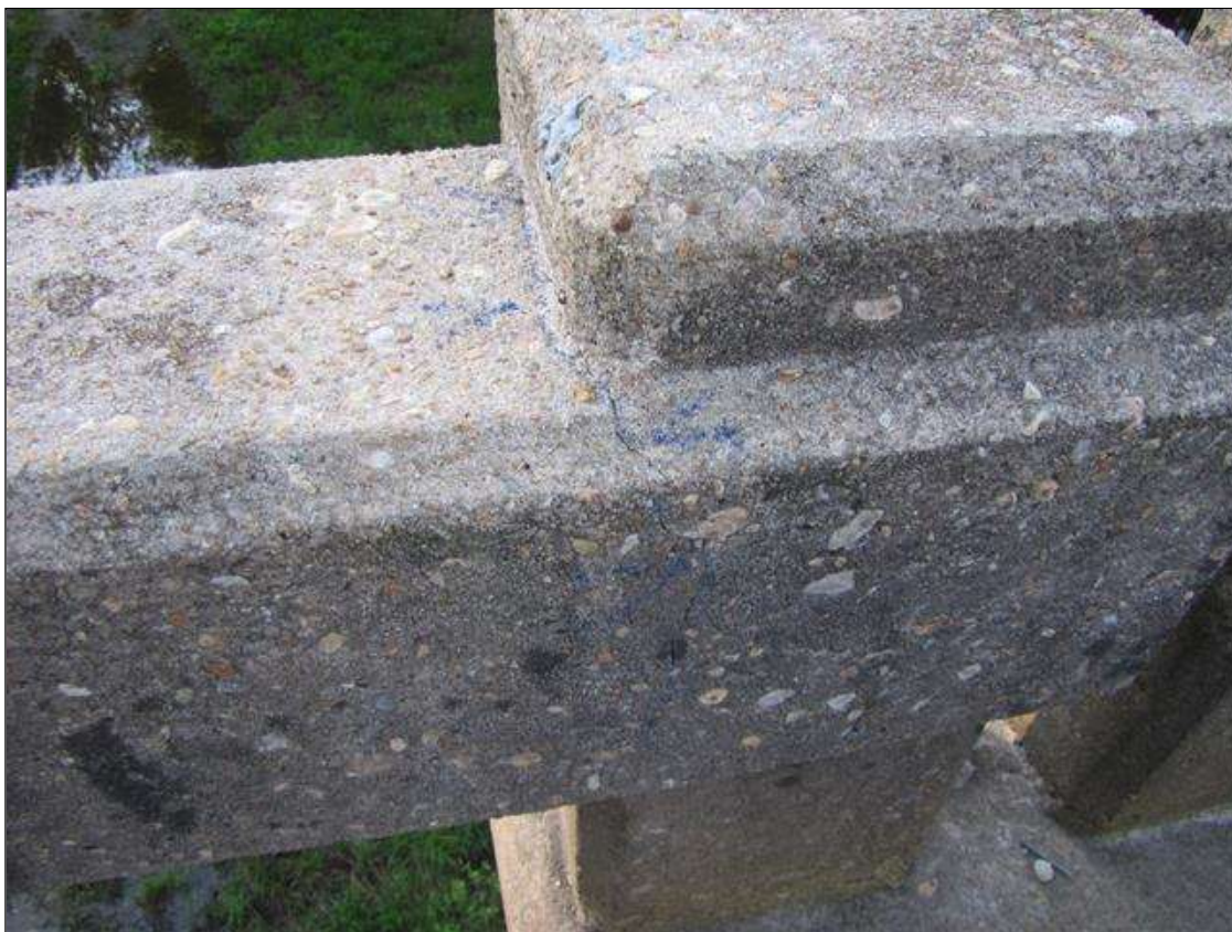
Span 3 Right Bridge Rail: (5) x up to 1/64" vertical and transverse cracks on concrete rail and curb (PHOTO TAKEN NEAR MIDSPAN)
