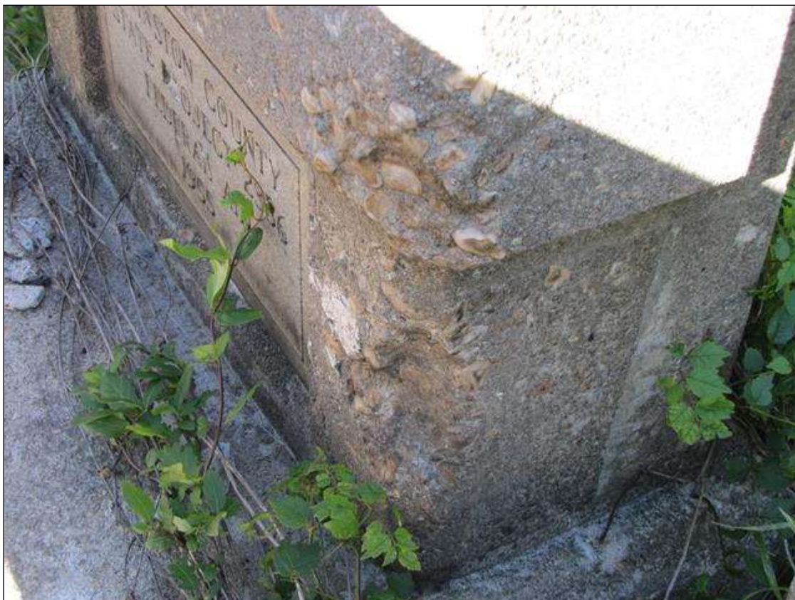
Span 4 Left Bridge Rail: (2) up to 3" x 5" x 1" deep spalls on end post
