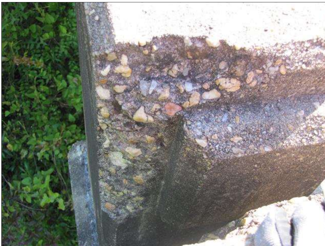
Span 4 Left Bridge Rail: 2" x 10" x 6" deep spall on concrete Post 7
