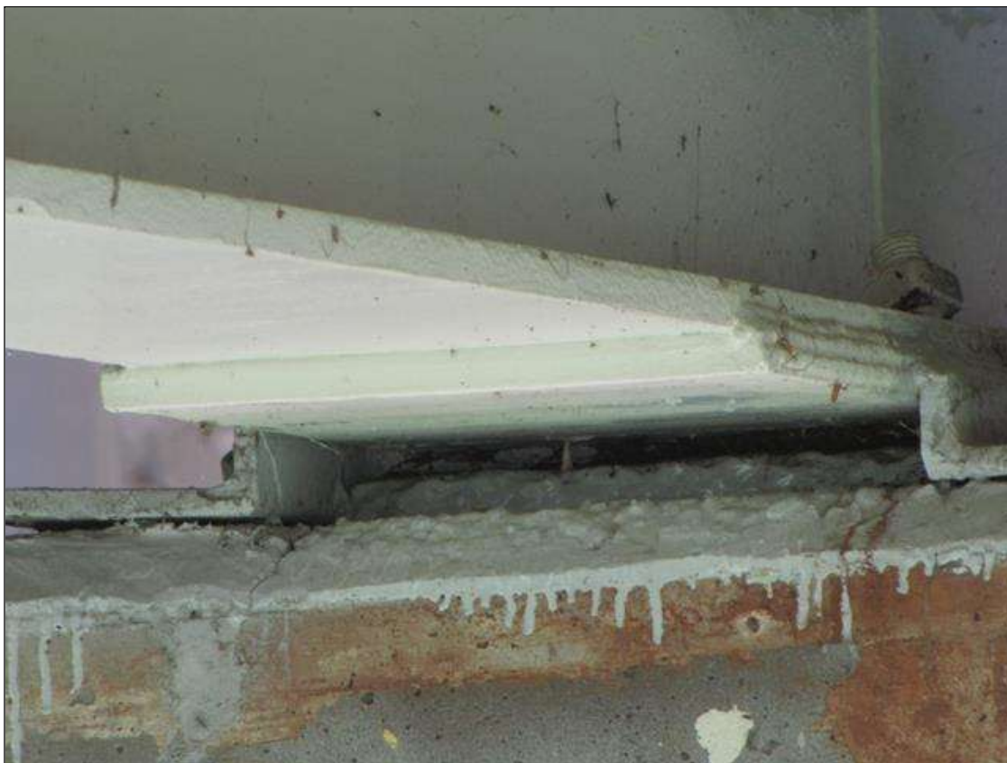
Span 1 Beam 2: 20" x 12" X 3/8" plate welded to bottom flange at Bent 1 (similar span 2 beam 2 at bent 1)
