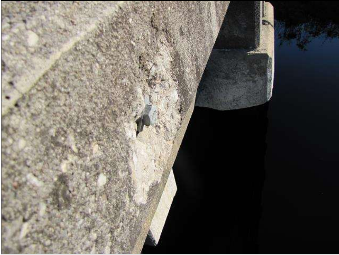
Span 1 Right Bridge Rail: 2- UP TO 7" x 6" x 1" spall on outside face of rail NEAR BENT 1
