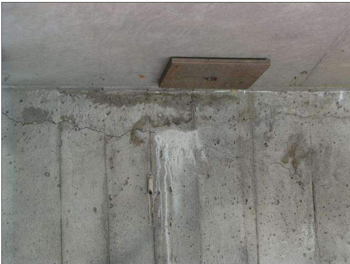
End Bent 2 Abutment/Backwall : 7' x up to 1/16" horizontal crack with efflorescence in Bay 3
