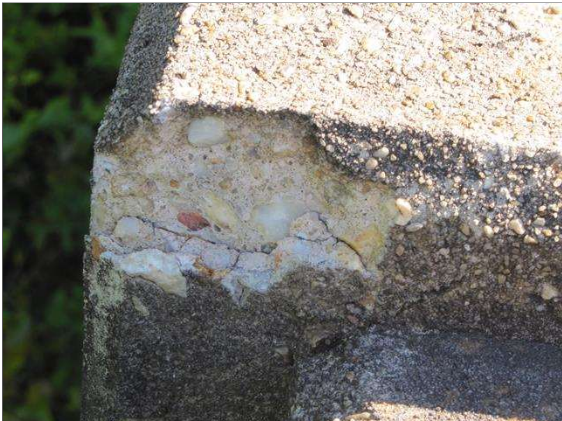
Span 4 Left Bridge Rail: 1" x 4" x 2" deep spall on concrete Post 6
