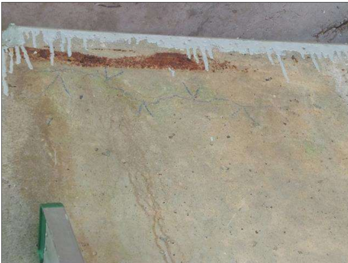
Bent 3 Cap 1: VERTICAL AND HORIZONTAL CRACKS UP TO 1/32" AT RANDOM THROUGHOUT (PHOTO TAKEN SOUTH FACE UNDER BEAM 2)
