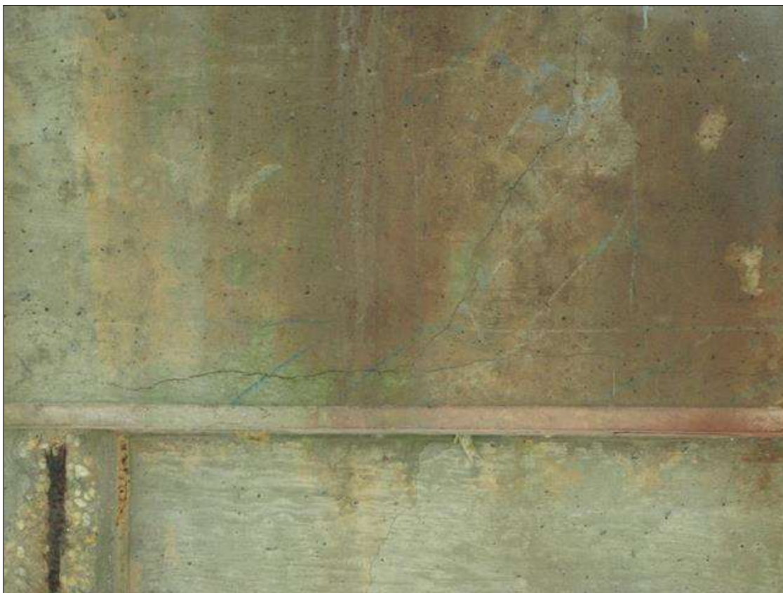
Bent 1 Cap 1: 42" x 24" area of hairline vertical and horizontal cracks on Span 1 face under Bay 1
