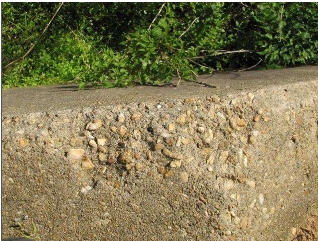
Wingwalls: 2 - 14" x 5" x 1" SPALLS ON TOP OF SOUTHEAST WINGWALL
