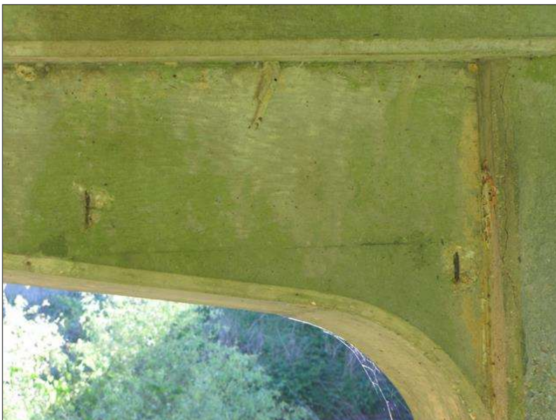
Bent 1 Pile 2: 2- UP TO 3" DIAMETER x 1/2" deep spall with exposed rebar on Span 1 face of corbel
