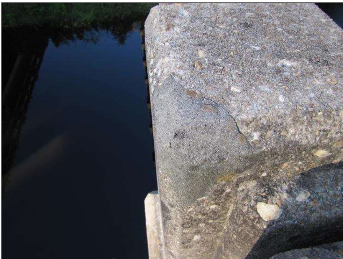
Span 2 Right Bridge Rail: 4" x 3" area of sound patch on top of Post 9
