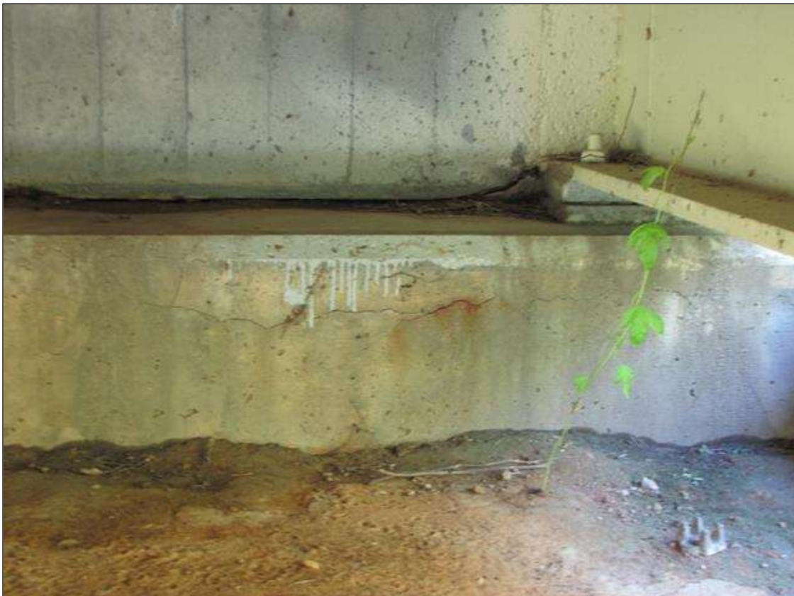
End Bent 1 Cap 1: 5' up to 1/32" horizontal crack WITH RUST STAINING under Bay 1
