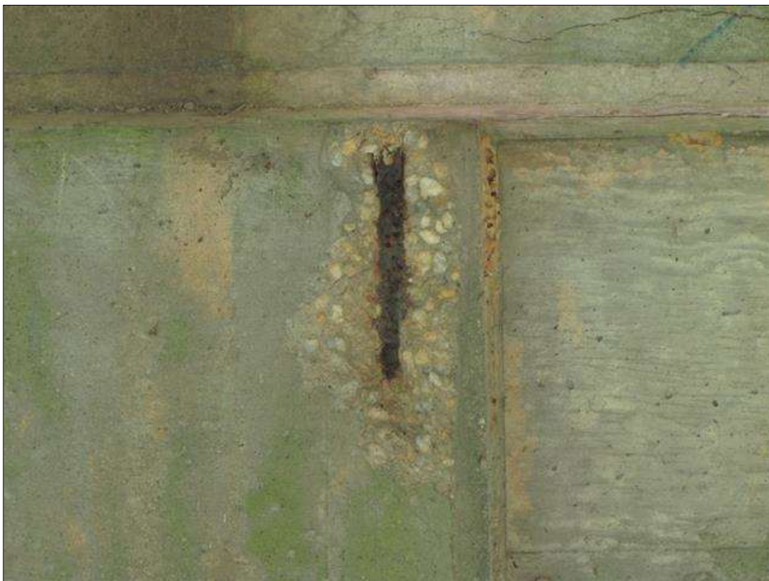
Bent 1 Pile 1: (PAR) 12" x 5" x 1" SPALL WITH EXPOSED REBAR ON SOUTH FACE AT BOTTOM OF CAP.
