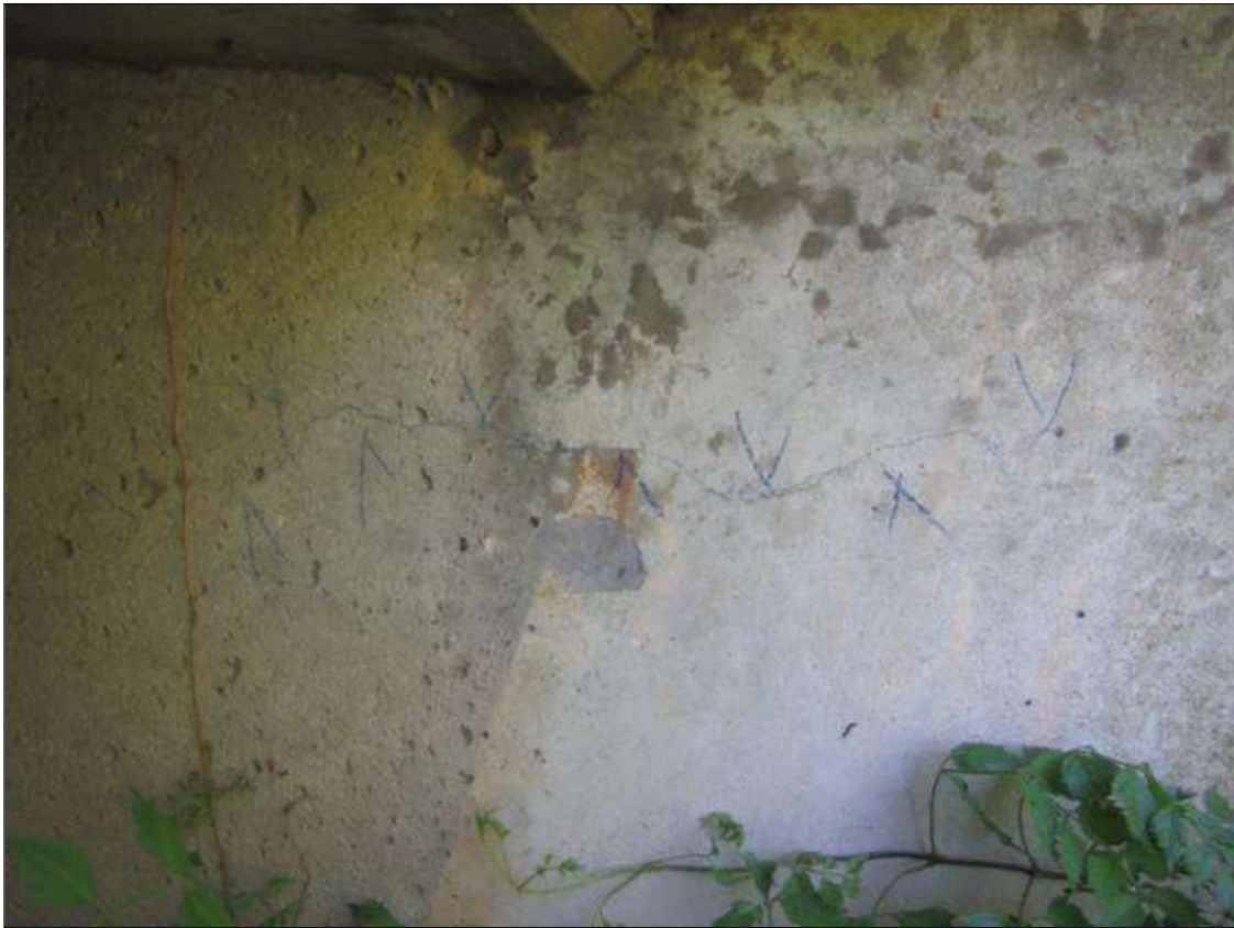
End Bent 1 Abutment/Backwall : 28" x up to 1/64" horizontal crack at West end
