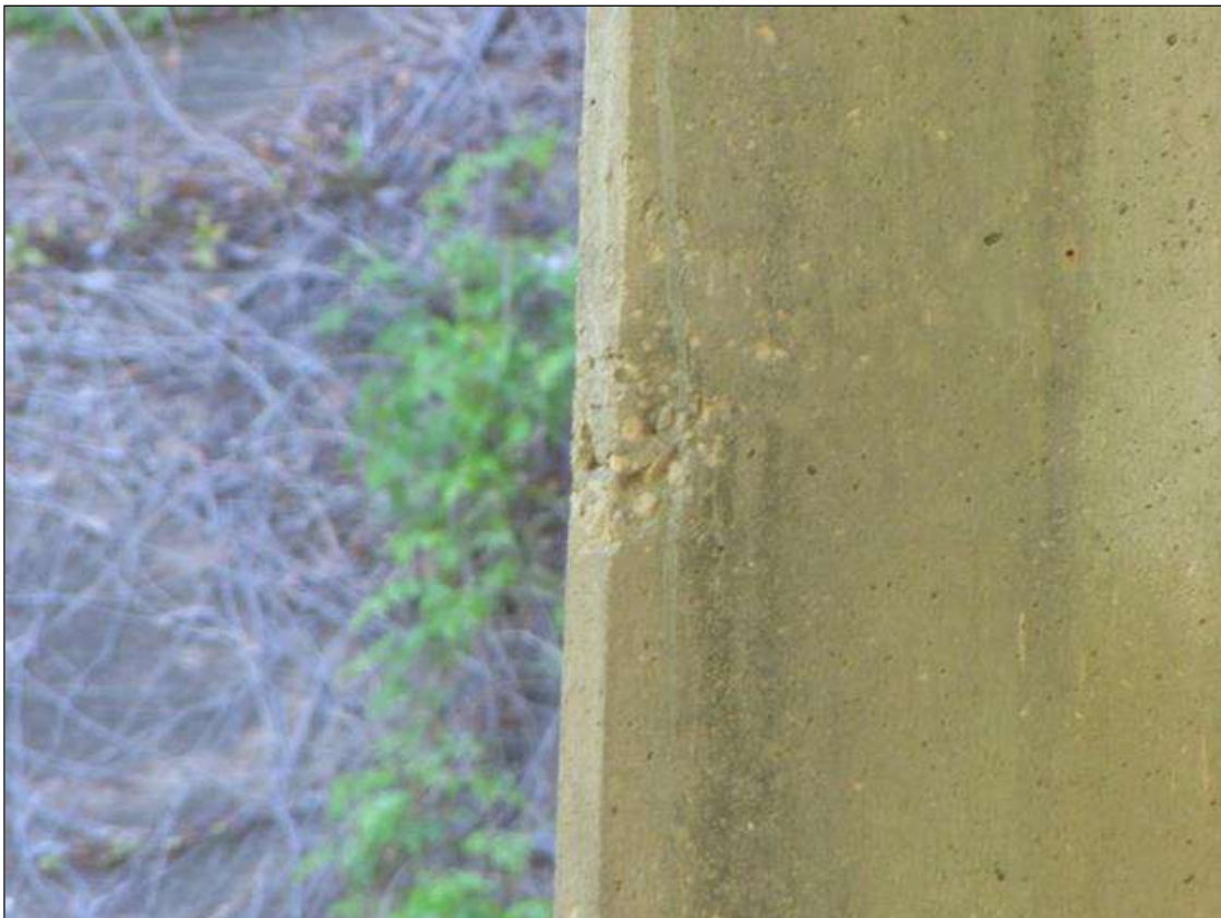
Bent 2 Pile 1: 4" x 2" area of honeycombing on SOUTHWEST corner 5' FROM BOTTOM OF CAP
