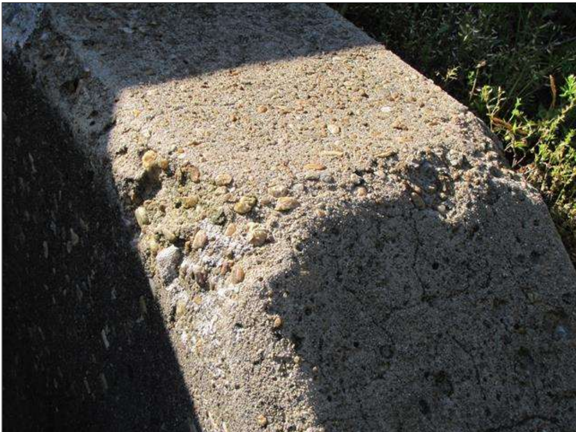
Wingwalls: 2 - UP TO 6" x 3" x 1" SPALLS ON TOP OF SOUTHWEST WINGWALL
