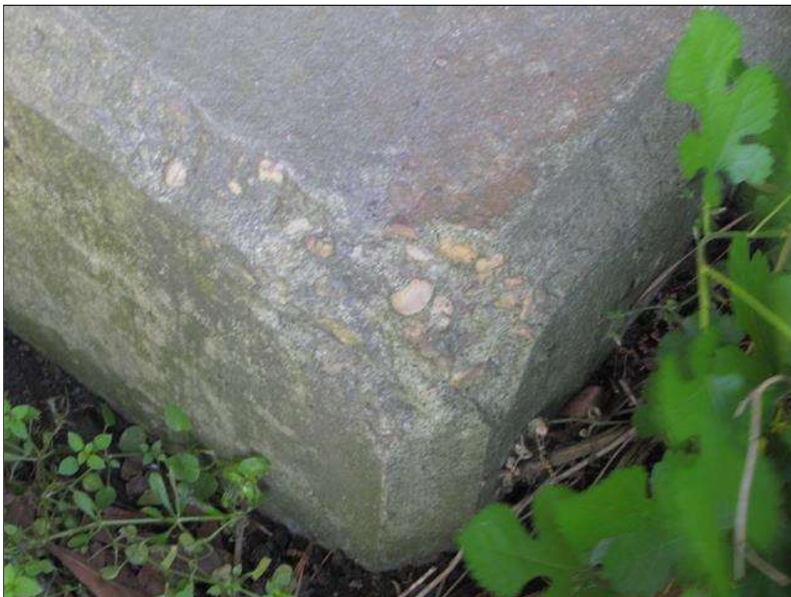
End Bent 1 Cap 1: 4" x 4" x 2" deep spall on Pile Cap 1
