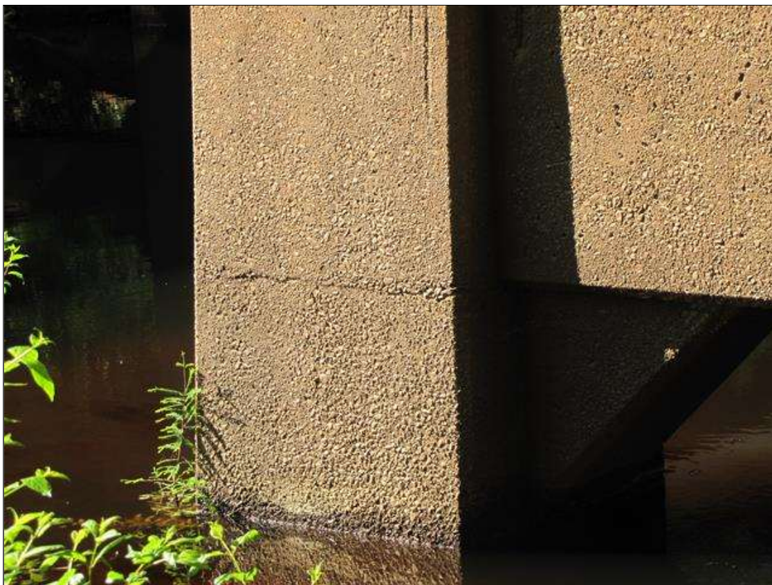
Bent 2 Pile 2: 4' ABRASION/WEAR 15' FROM BOTTOM OF CAP
