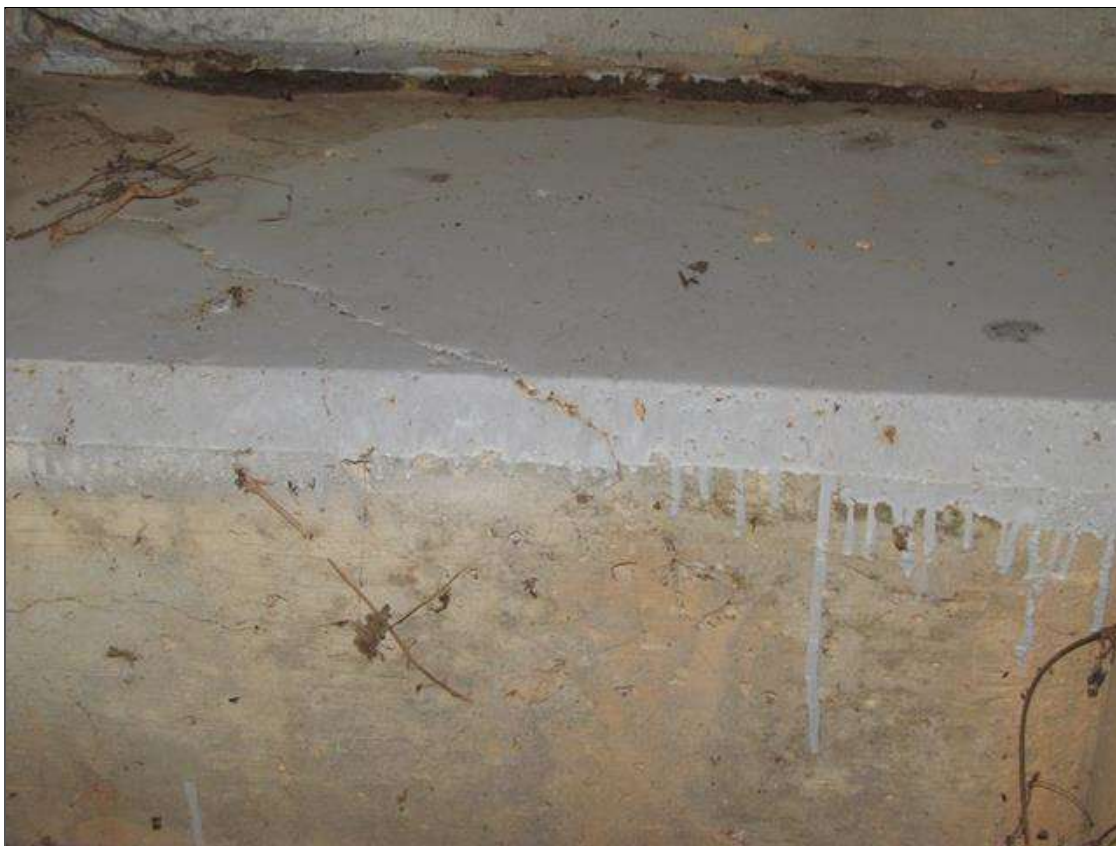
End Bent 1 Cap 1: 6' x 1/16" horizontal crack under Bay 2
