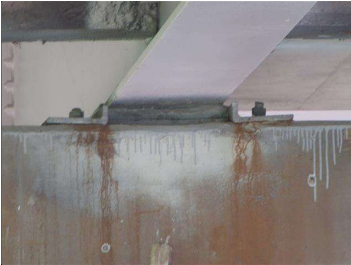
Bent 2 Cap 1: 4' x 15" area of sound patch on Span 2 face under Beam 3 (Beam 2 similar)
