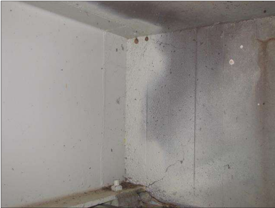
Span 1 Beam 3: 7" x 31" REPAIR AT END BENT 1
