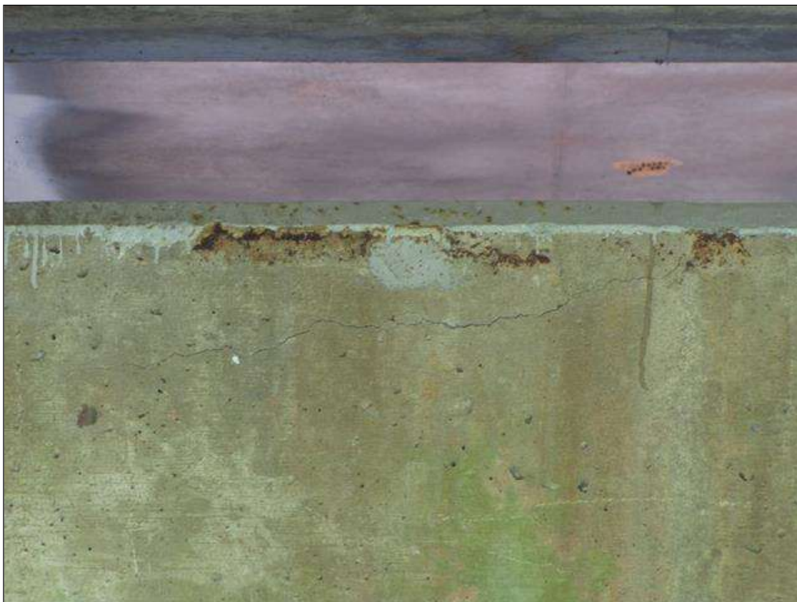
Bent 1 Cap 1: 2' X UP TO 1/32" HORIZONTAL CRACK UNDER BAY 2 NEAR TOP SOUTH FACE
