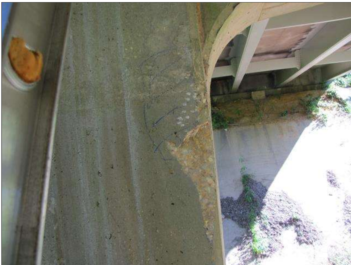
Bent 3 Pile 1: 14" X UP TO 6" X 2" SPALL WITH ADJACENT 1' DIAMETER DELAMINATION ON SOUTHEAST CORNER 2' FROM BOTTOM OF CAP.
