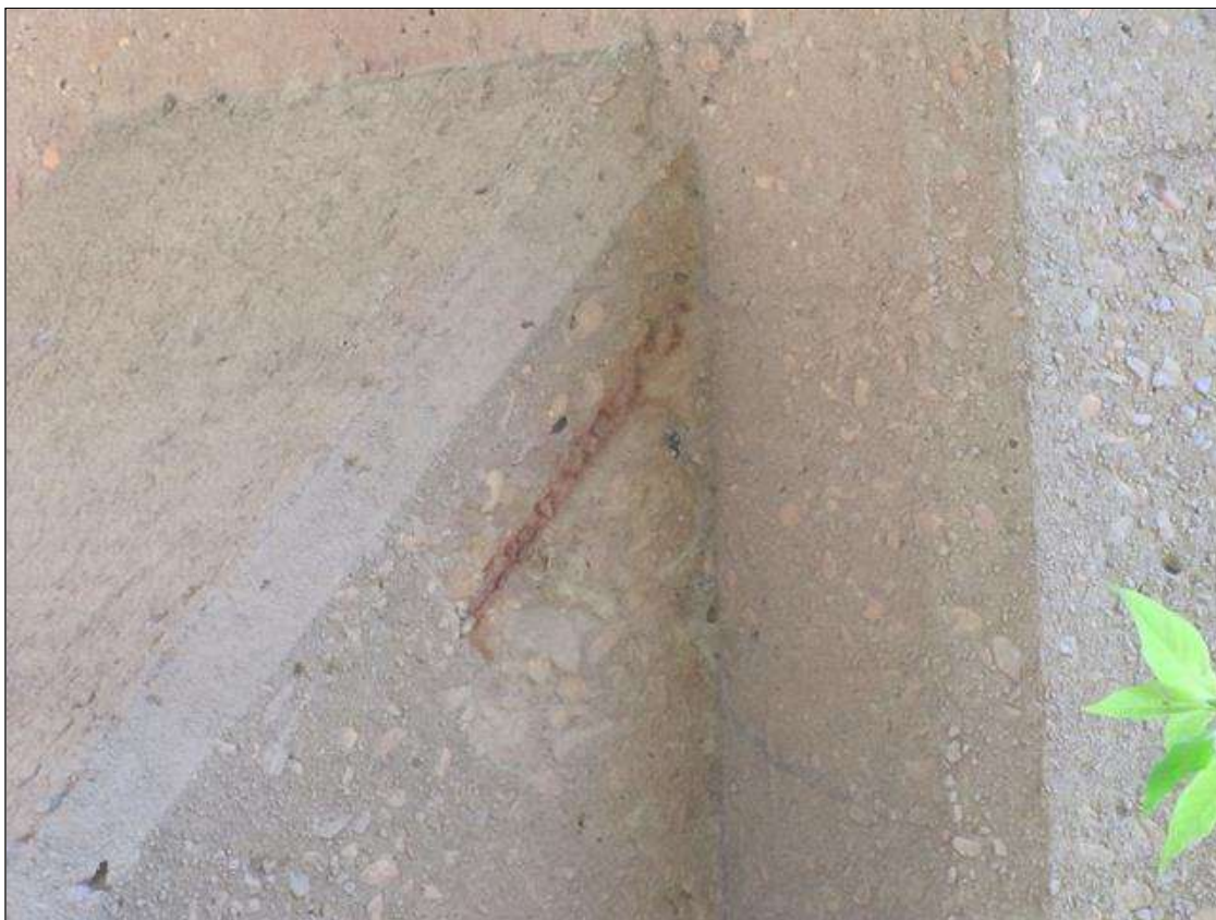
Bent 3 Pile 2: 6" x 8" x 1" deep spall with exposed rebar on Span 3 face of corbel above strut
