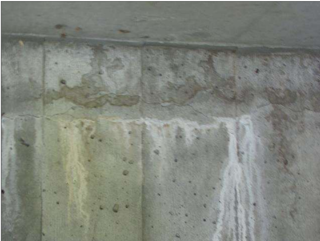
End Bent 1 Abutment/Backwall : 6' x up to 1/64" horizontal crack WITH EFFLORESCENCE in Bay 1 (Bays 2 and 3 similar)
