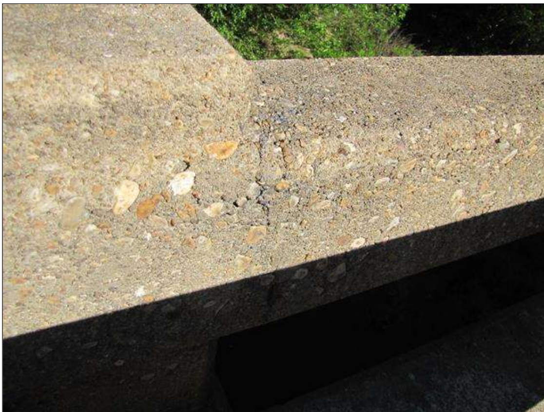
Span 2 Left Bridge Rail: (4) x up to 1/64" vertical and transverse cracks on concrete rail and curb
