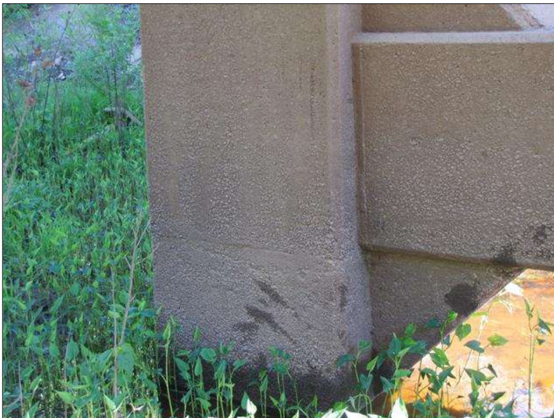
Bent 3 Pile 1: 3' ABRASION/WEAR 15' FROM BOTTOM OF CAP
