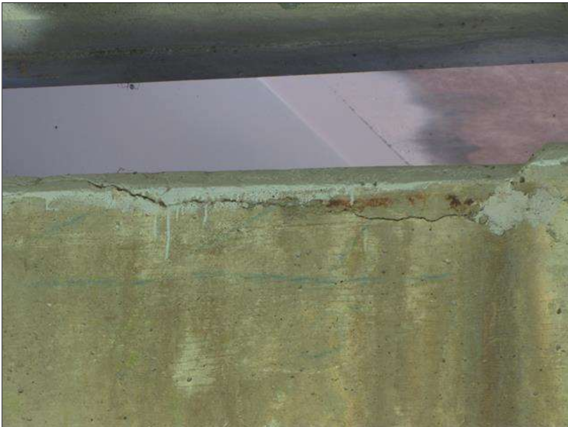
Bent 1 Cap 1: 18" up to 1/8" horizontal crack on Span 1 face under Bay 1
