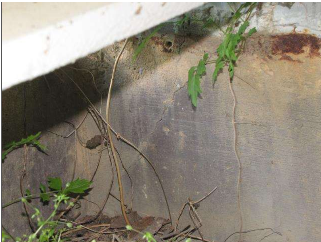
End Bent 1 Cap 1: 16" up to 1/16" diagonal crack under Beam 4 (Beam 1 similar)
