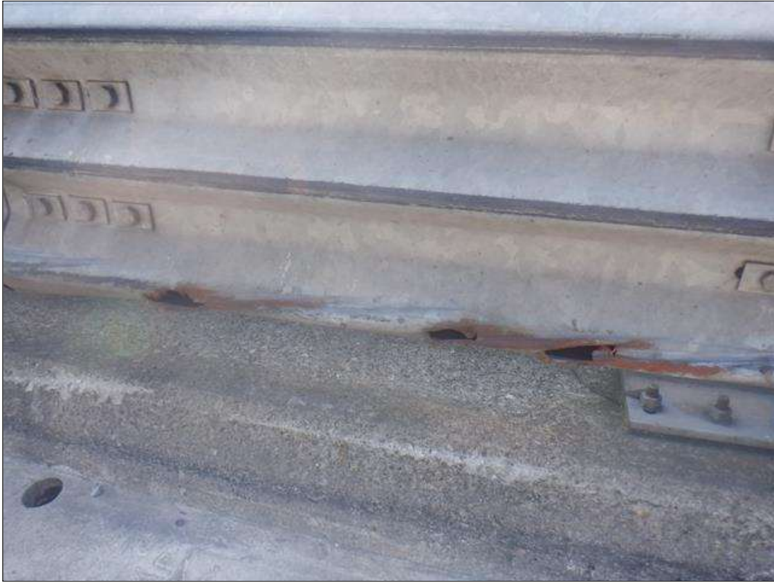
Span 8 Right Bridge Rail: HEAVY IMPACT DAMAGE WITH UP TO 3 IN LONG X 1 IN HIGH HOLES AND DENTS IN THE BOTTOM OF SUPPLMENTAL BRIDGE RAIL FOR FULL SPAN LENGTH. DAMAGE EXTENDS INTO SPANS 7 AND 6.
