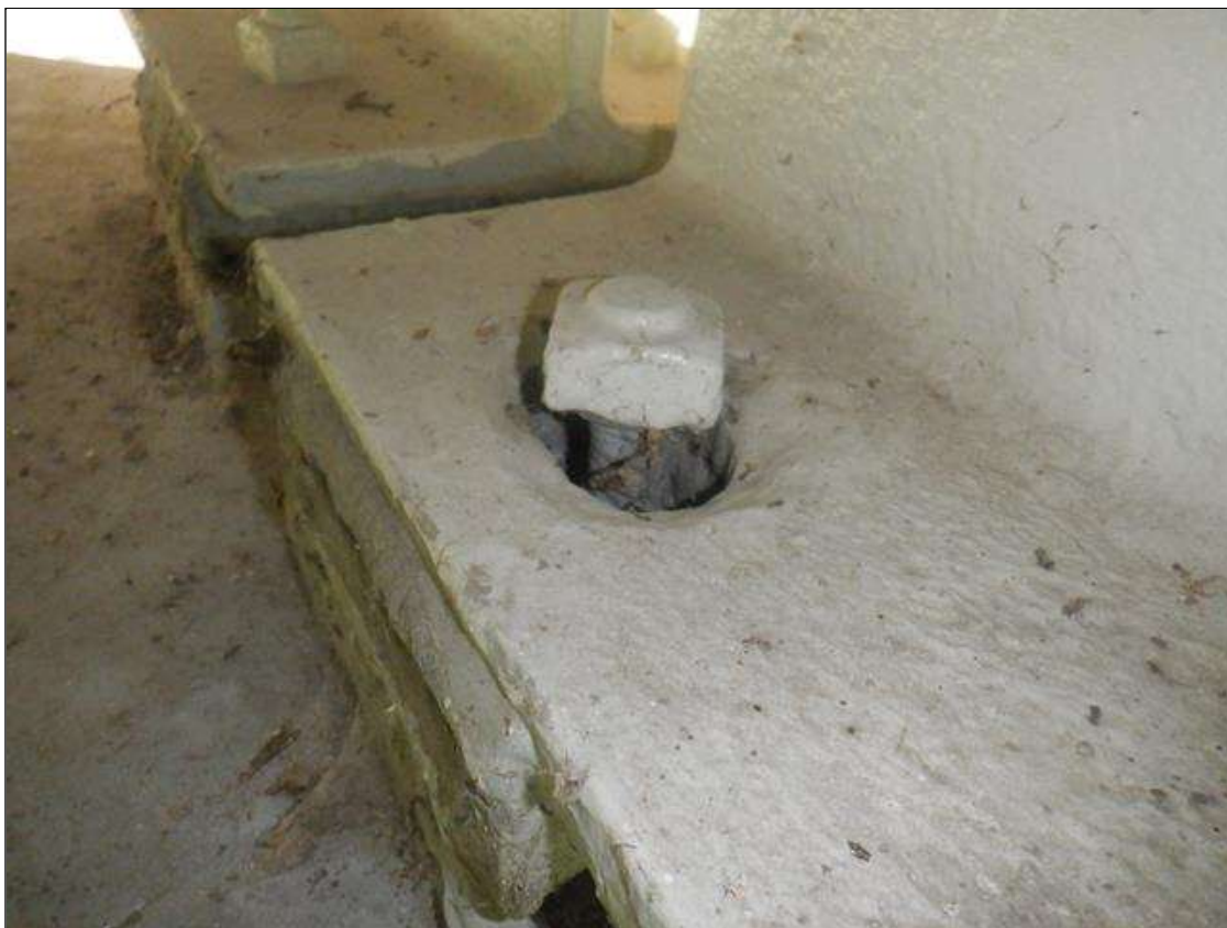
Span 3 Far Bearing: ANCHOR BOLT NUT NOT CONNECTED COMPLETELY
