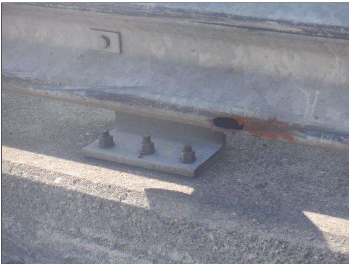
Span 2 Right Bridge Rail: IMPACT DAMAGE WITH SCRAPE MARKS FOR FULL SPAN LENTH IN BOTTOM OF SUPPLEMENTAL RAIL.
