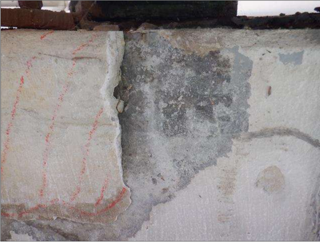
Span 4 Beam 3 - Far Bearing: NEW BEARING HAS A LOSS OF BEARING AREA DUE TO SPALL ON CAP. AREA REPAIRED IS UNSOUND AND HAS 6 IN HIGH X 5 IN WIDE X 2 IN DEEP SPALLS. (PAR)
