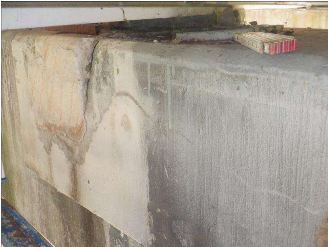
Bent 4 Cap 1: 3.5 FT LONG X 1.5 FT HIGH UNSOUND PATCHED AREA WITH SPALLS, TOP OF SOUTH FACE, BELOW BEAM 3.
