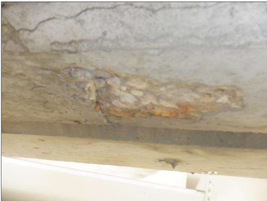
Span 5 Deck: 6 IN DIAMETER X 3/4 IN DEEP SPALL IN INTERMEDIATE DIAPHRAGM IN BAY 2 ABOVE BENT 5.
