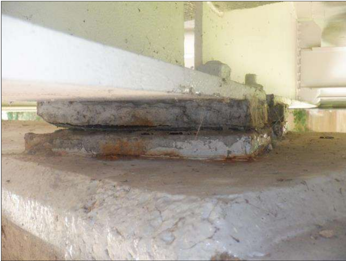
Span 6 Far Bearing: BEARINGS HAVE BEEN PAINTED SINCE PREVIOUS INSPECTION. SECTION LOSS EXISTS BENEATH THE PAINTED SURFACES IN BOTH MASONRY AND SOLE PLATES. UP TO 90% SECTION REMAINING.
