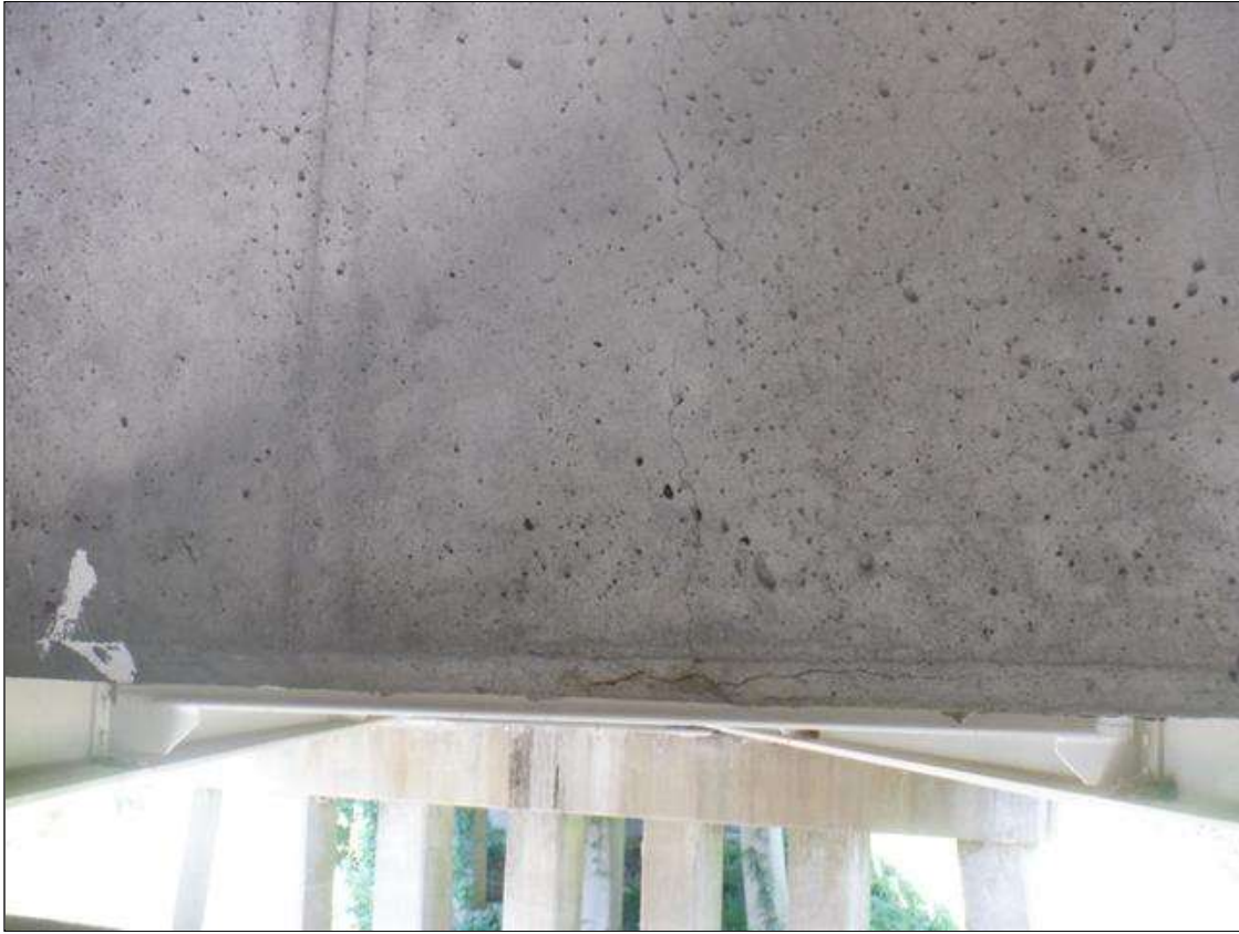
Span 5 Deck: UP TO 0.05 IN WIDE X 2 FT HIGH VERTICAL CRACKS IN BENT DIAPHRAGM IN SEVERAL BAYS AT BENT 5
