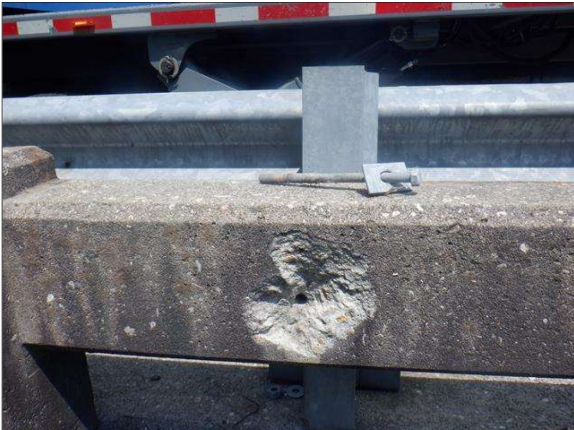
Span 2 Right Bridge Rail: BOLT HAS DETACHED FROM CONCRETE OUTER RAIL 10 FT FROM END BENT 1 LEAVING METAL INNER RAIL FREE. (PAR)
