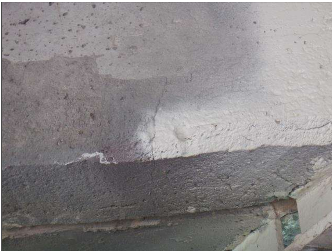
Span 4 Deck: 4 FT LONG X 1 FT HIGH AREA OF UNSOUND CONCRETE PATCH WITH UP TO 0.05 IN VERTICAL CRACKS IN BAY 3 BENT DIAPHRAGM AT BENT BENT 3
