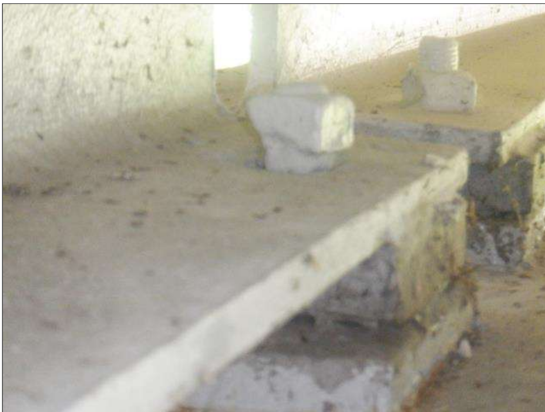
Span 6 Far Bearing: LEFT ANCHOR BOLT HAS UP TO 80% SECTION REMAINING AND ANCHOR BOLT NUT HAS UP TO 50% SECTION REMAINING.
