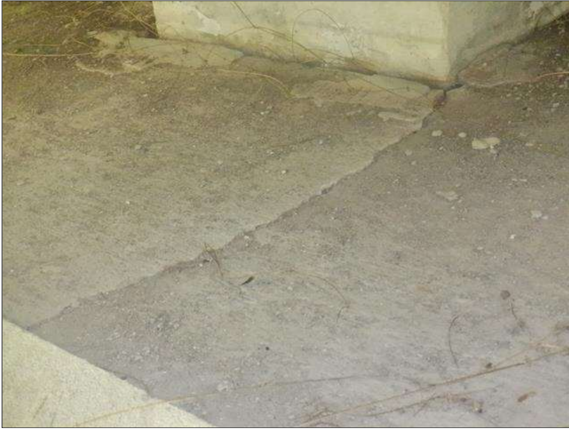
UP 3 FT LONG X 1/4 IN WIDE LONGITUDINAL CRACK IN TOP OF SLOPE PROTECTION AT BAY 2, IN BENT 1
