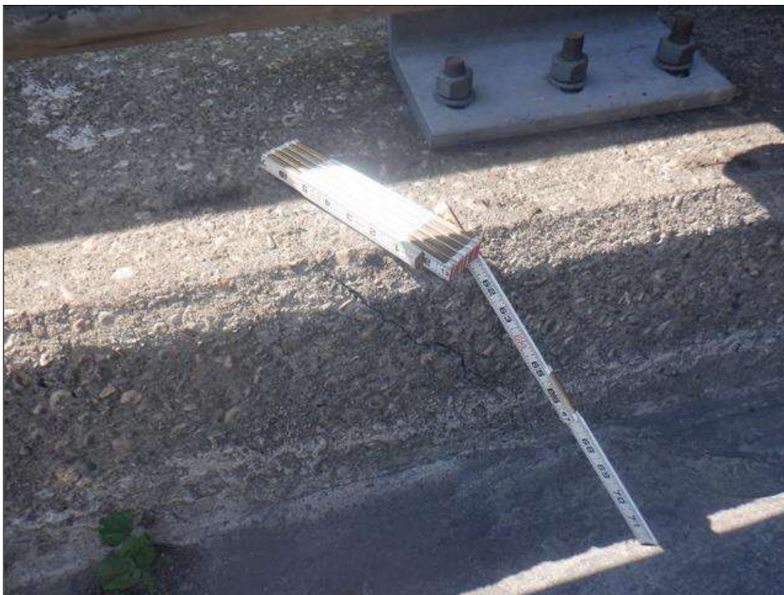
Span 2 Right Bridge Rail: UP TO 0.03 IN WIDE X 2 FT LONG DIAGONAL CRACKS IN BOTTOM OF CURB AT 1 FT FROM BENT 2.
