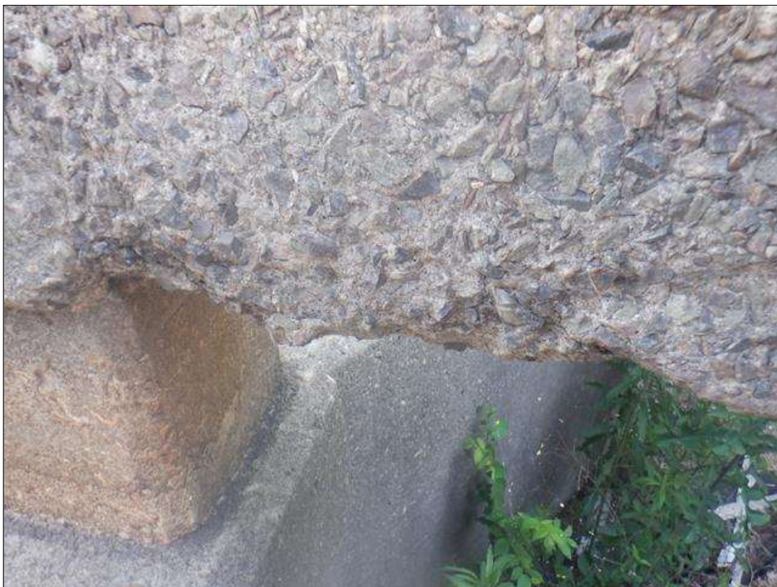
Span 8 Right Bridge Rail: 1 FT LONG X 4 IN WIDE X 1 IN DEEP SPALL IN BOTTOM FACE AT END BENT 2
