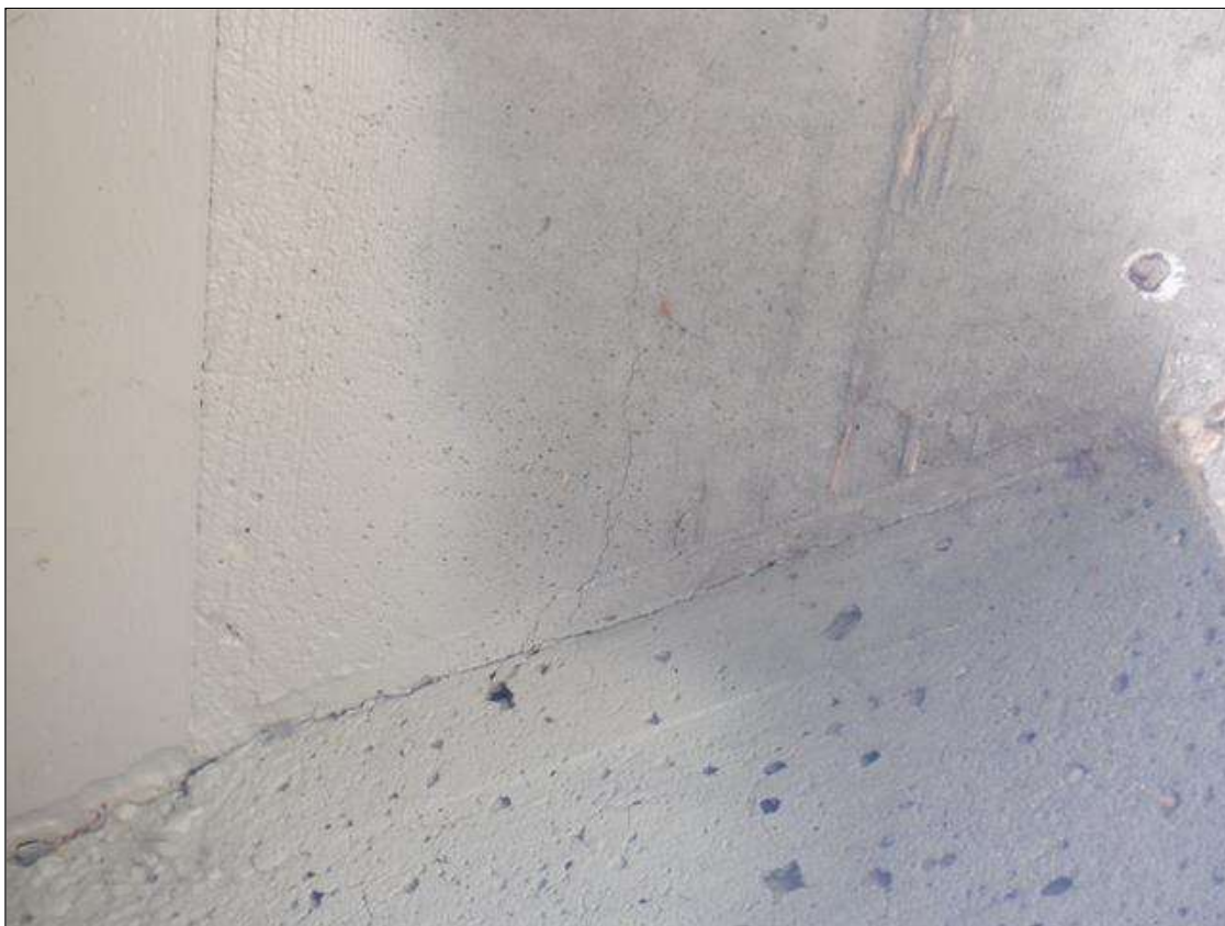
Span 4 Deck: EIGHT (8) UP TO 0.02 IN WIDE X UP TO 3 FT LONG TRANSVERSE CRACKS IN LEFT OVERHANG.
