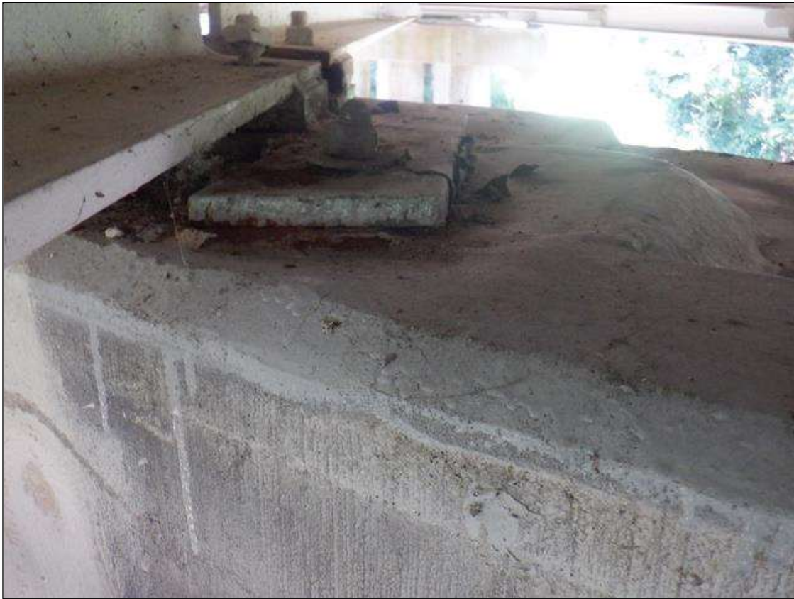
Bent 4 Cap 1: NEW REPAIR 18 IN WIDE X 1 FT HIGH UNSOUND CONCRETE PATCH IN SOUTH FACE BELOW BEAM 3. BEARING IS NOT SEATED LEVEL. REPAIRS MADE SINCE PREVIOUS INSPECTION ARE UNSOUND
