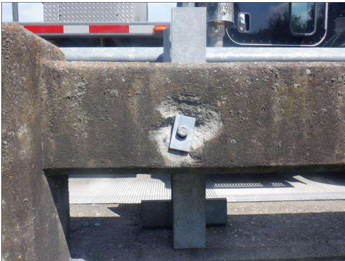
Span 1 Right Bridge Rail: UP TO 6 IN DIAMETER X 1.5 IN DEEP SPALL IN EXTERIOR FACE AT ANCHOR BOLT CONNECTION. TYPICAL AT SEVERAL CONNECTIONS.
