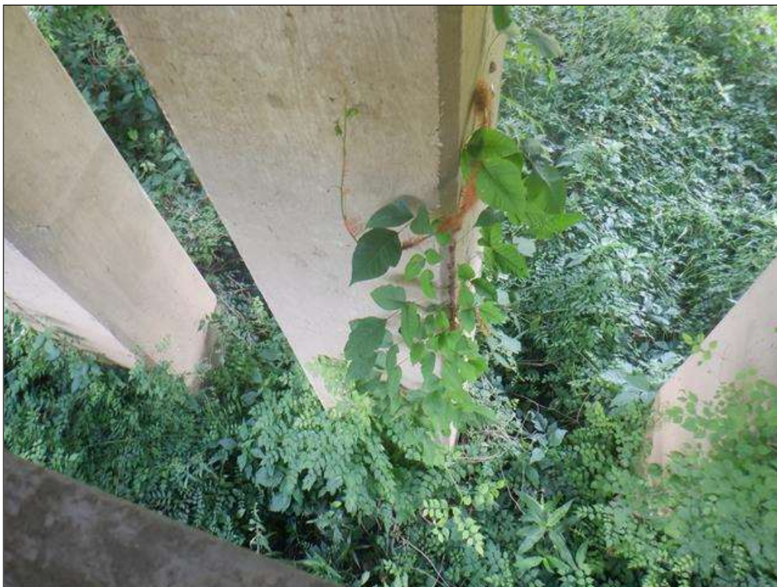
Bent 1 Pile 3: MINOR VEGETATION GROWTH IN SOUTH AND NORTH FACES.
