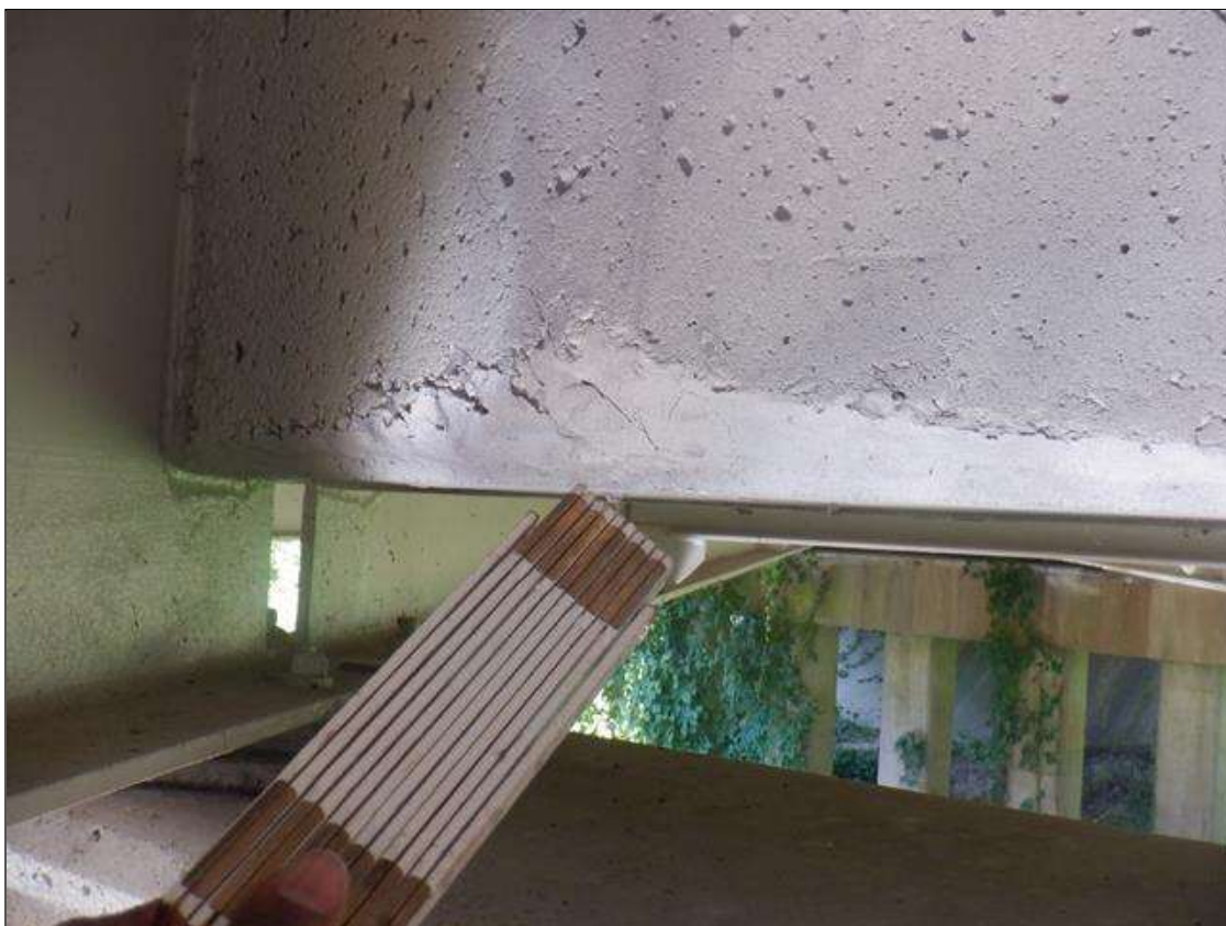
Span 6 Deck: 38 IN LONG X 1 FT HIGH SOUND CONCRETE PATCHED AREA, BOTTOM OF BAY 2 END DIAPHRAGM, AT BENT 6.
