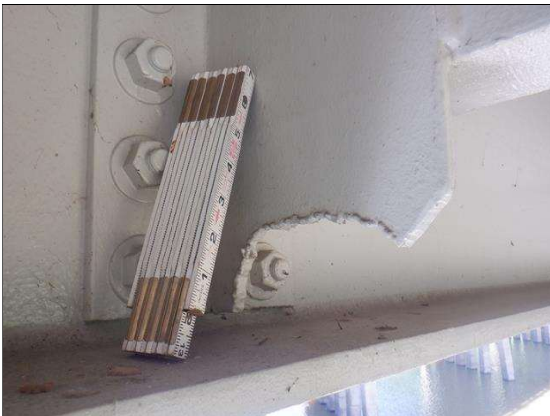
Span 4 Beam 1: 2 IN HIGH OF INTERMEDIATE STIFFENER IS CUT OUT AT BOTTOM AT BOTH LOCATIONS. PAR IS NOT ISSUED AS IT APPEARS TO BE FROM PREVIOUS BRIDGE REPAIR.
