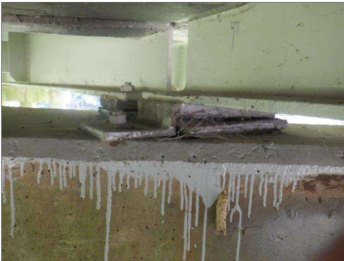
Span 1 Far Bearing: WELDED REPAIR WITH NEW ANCHOR BOLT.
