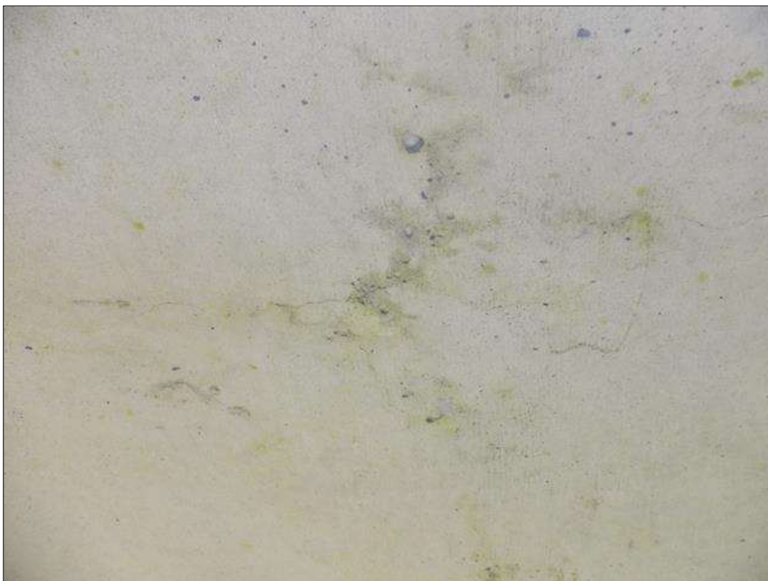
Span 3 Deck: UP TO 0.03 IN WIDE RANDOM CRACKING IN DECK UNDERSIDE, SCATTERED THROUGHOUT.
