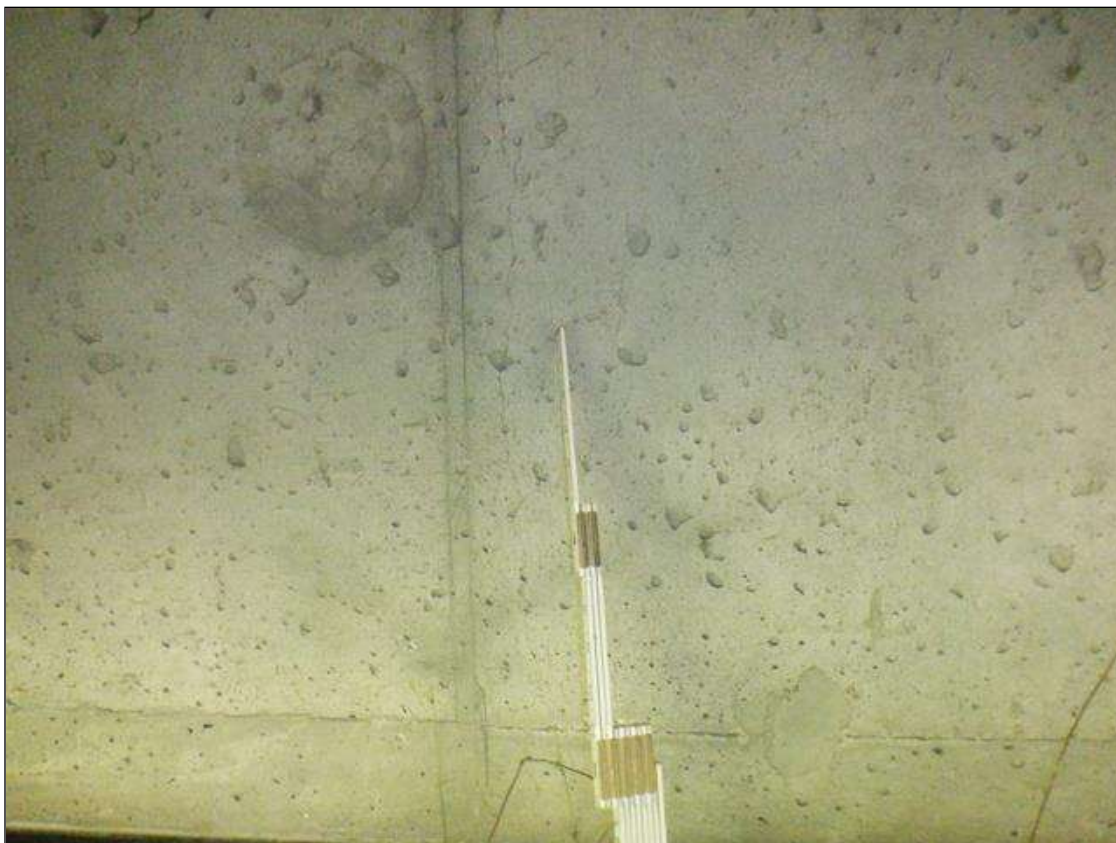
End Bent 2 Abutment: 4 FT HIGH X UP TO 0.05 IN WIDE VERTICAL CRACK IN BAY 2
