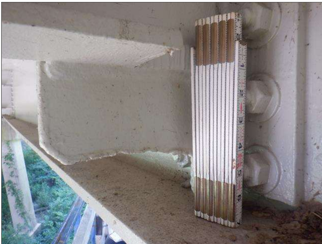
Span 7 Beam 4: 2 IN HIGH OF INTERMEDIATE STIFFENER IS CUT OUT AT BOTTOM AT BOTH LOCATIONS. PAR IS NOT ISSUED AS IT APPEARS TO BE FROM PREVIOUS BRIDGE REPAIR.
