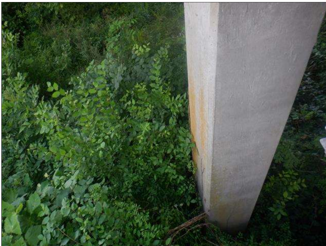
Bent 1 Pile 1: VEGETATION GROWTH ALONG SOUTHWEST CORNER FOR UP TO 12 FT HIGH.
