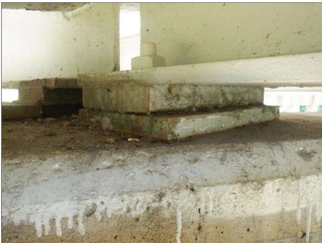
Span 4 Beam 3 - Near Bearing - Protective System: NEW REPAIR: PROTECTIVE SYSTEM IS REPAINTED SINCE PREVIOUS INSPECTION.
