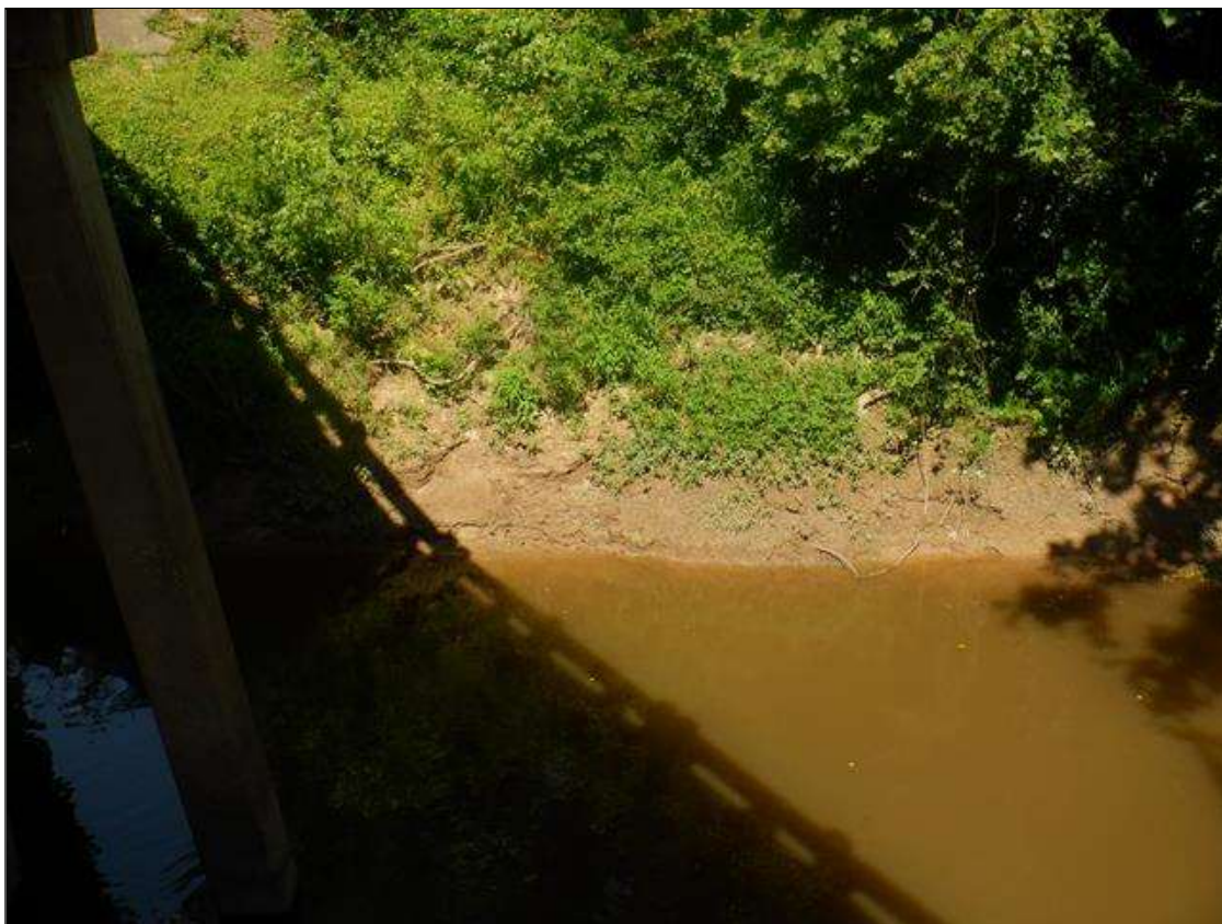
50 FT LONG X 4 FT HIGH X 4 FT DEEP AREA OF EROSION ALONG NORTH BANK
