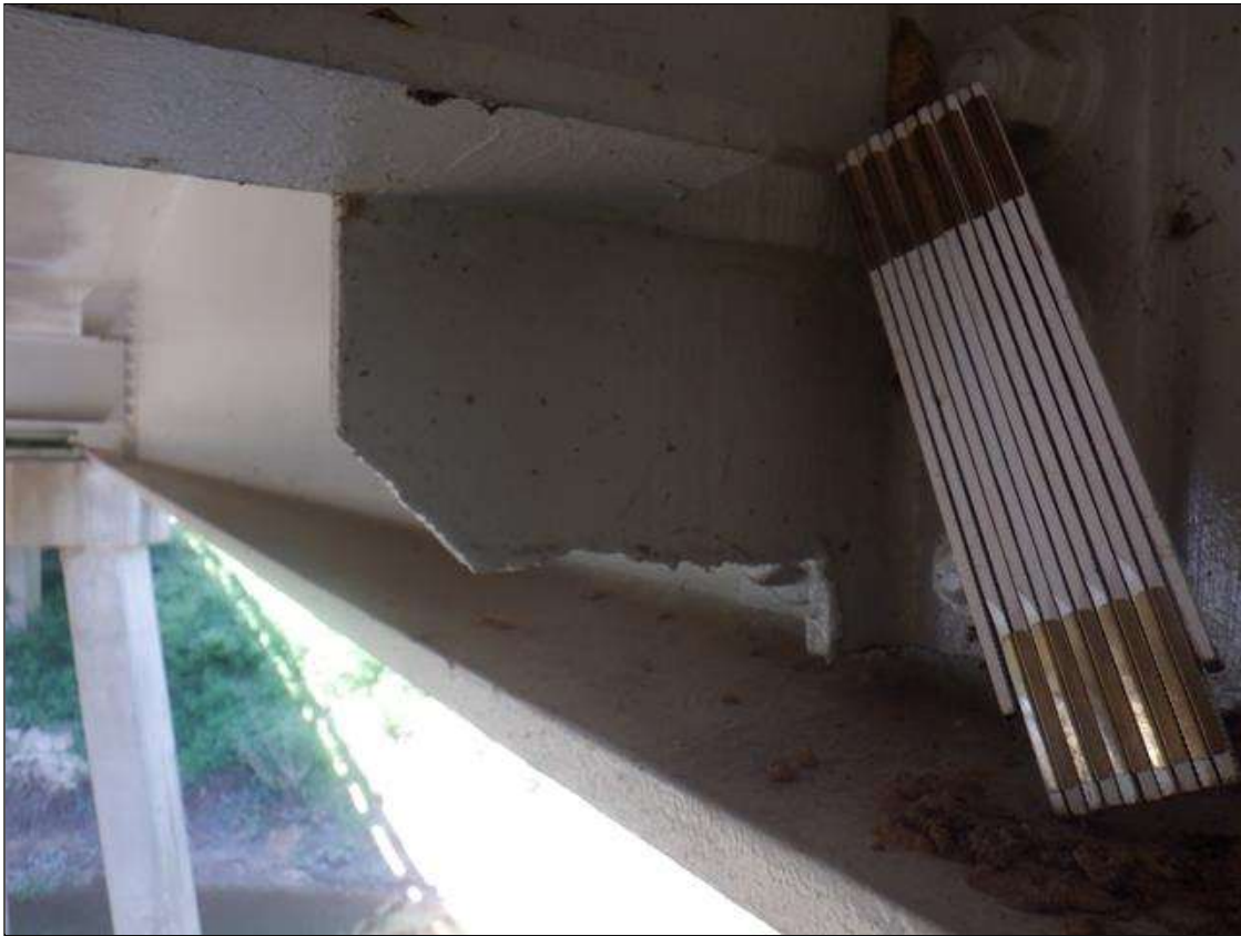
Span 6 Beam 4: 2 IN HIGH OF INTERMEDIATE STIFFENER IS CUT OUT AT BOTTOM AT BOTH LOCATIONS. PAR IS NOT ISSUED AS IT APPEARS TO BE FROM PREVIOUS BRIDGE REPAIR.
