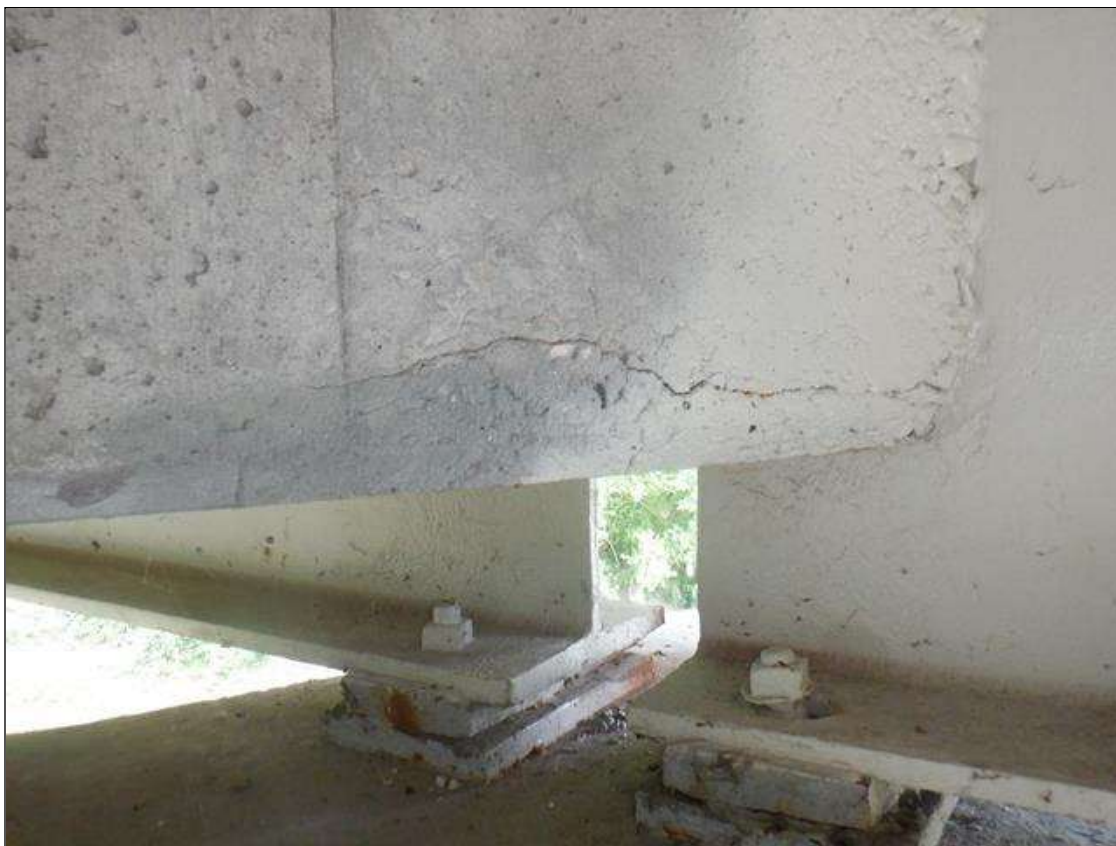
Span 5 Beam 4: 3 FT LONG X 1/16 IN WIDE HORIZONTAL CRACK IN BENT DIAPHRAGM AT BENT 5
