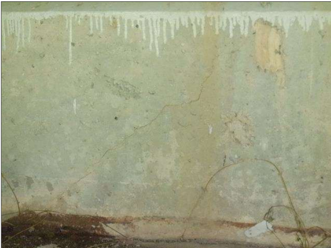
End Bent 1 Cap 1: TWO (2) 2 FT LONG X 0.03 IN WIDE DIAGONAL CRACKS IN FACE OF CAP BELOW BAY 2.
