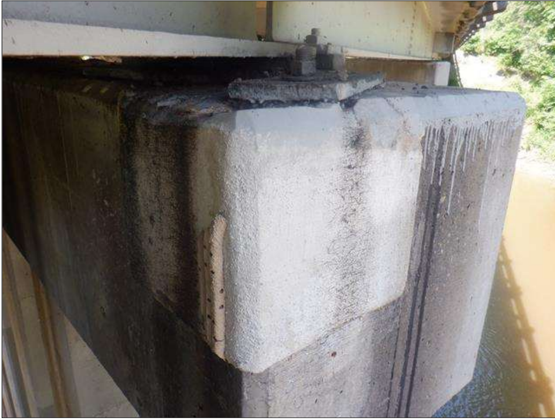
Bent 4 Cap 1: 15 IN HIGH X 21 IN WIDE SOUND CONCRETE PATCH AREA, TOP SOUTHEAST CORNER OF CAP, BELOW NEW BEARING ASSEMBLY OF BEAM 4. PATCH EXHIBITS A 8 IN LONG X 0.02 IN WIDE DIAGONAL CRACK STARTING AT TOP LEFT CORNER IN SOUTH FACE AND A UP TO 0.03 IN WIDE X 15 IN LONG VERTICAL CRACK IN EAST FACE.
