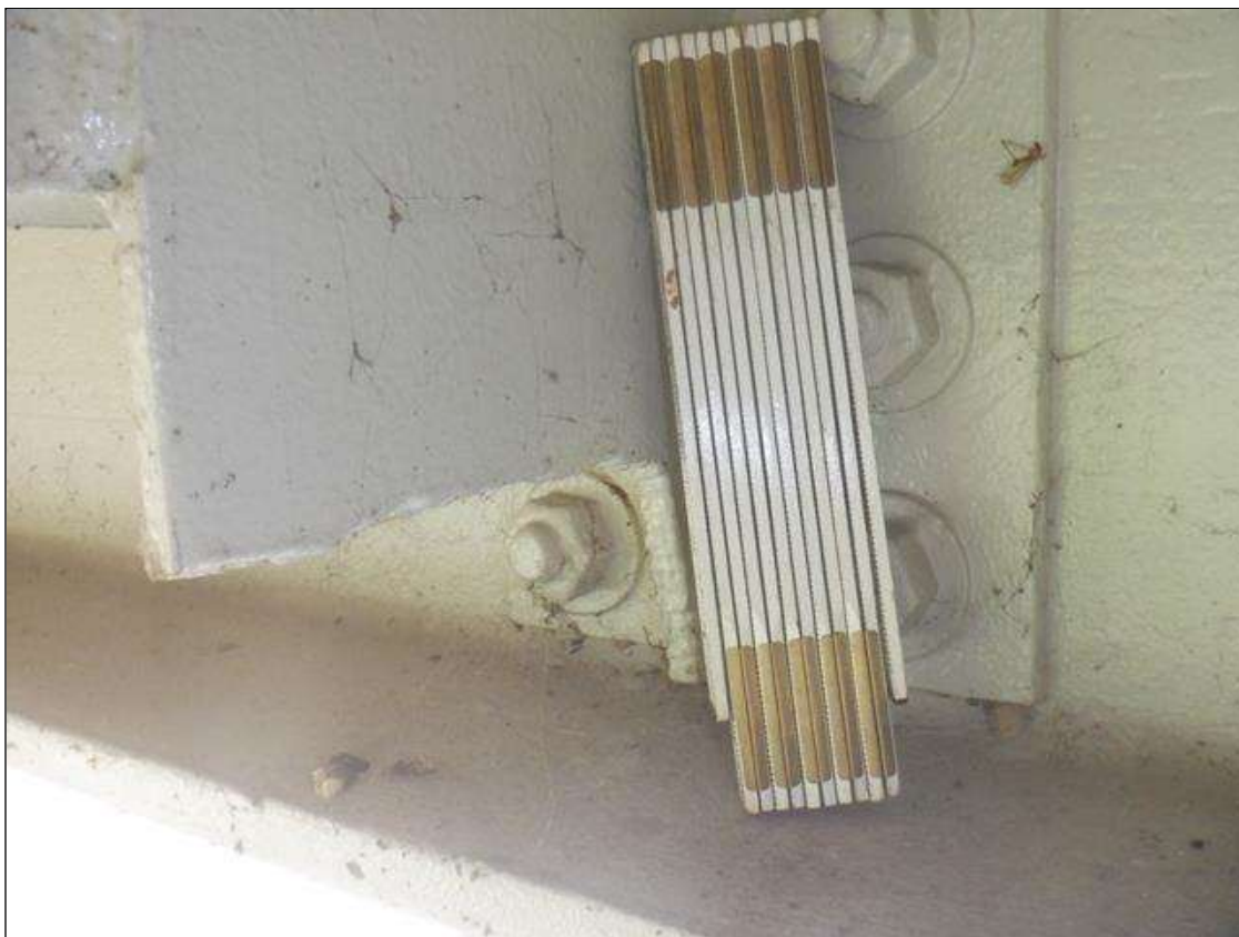
Span 3 Beam 4: 2 IN HIGH OF INTERMEDIATE STIFFENER IS CUT OUT AT BOTH LOCATIONS. PAR IS NOT ISSUED AS IT APPEARS TO BE FROM PREVIOUS BRIDGE REPAIR.
