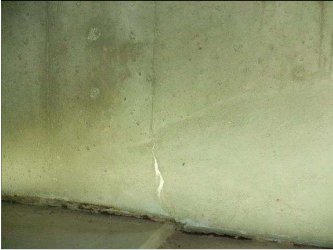
End Bent 1 Abutment: 3 FT HIGH X 0.05 IN WIDE VERTICAL CRACK WITH EFFLORESCENCE IN BAYS 1 AND 2
