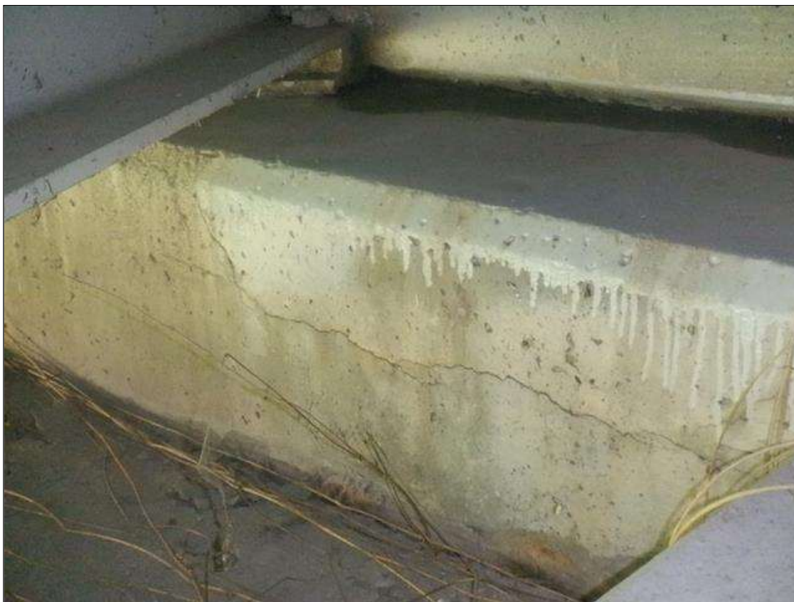
End Bent 2 Cap 1: 3 FT LONG X 1/16 IN WIDE HORIZONTAL CRACK, BELOW BEAM 2. TYPICAL AT BEAM 3.
