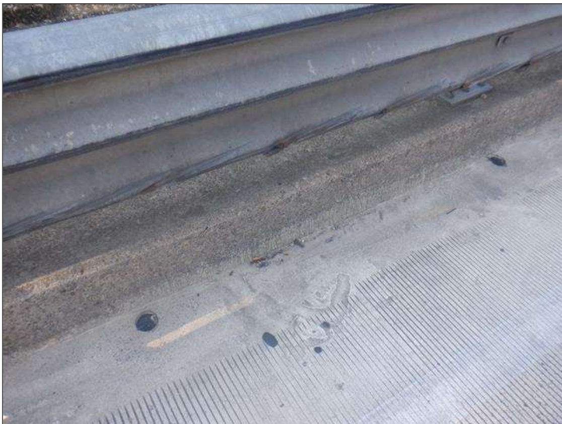
TYPICAL DRAINAGE HOLES ALONG RIGHT BRIDGE RAIL SIMILAR ALONG LEFT BRIDGE RAIL
