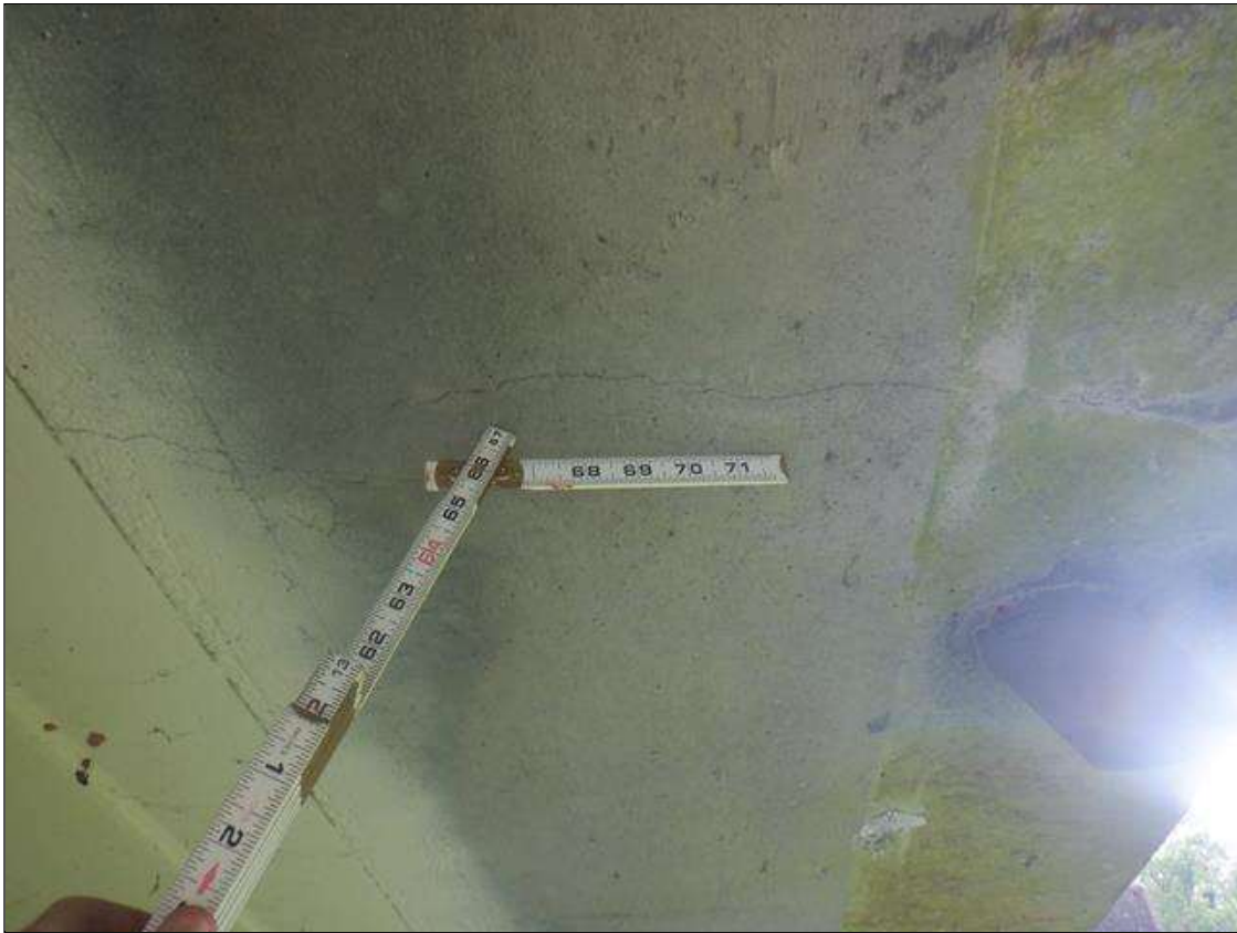
Span 2 Deck: NINE (9) UP TO 0.02 IN WIDE X UP TO 3 FT LONG TRANSVERSE CRACKS IN LEFT OVERHANG. TYPICAL AT RIGHT OVERHANG.
