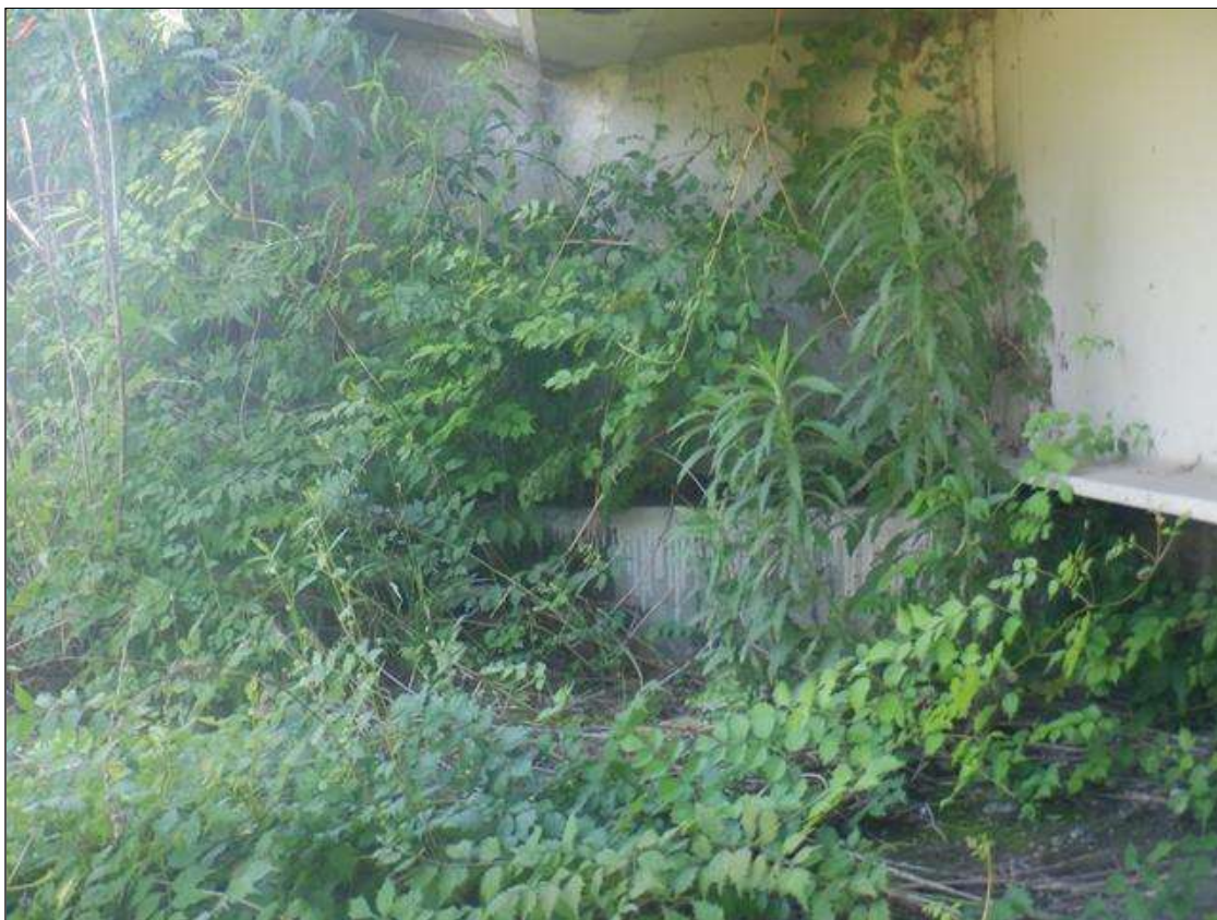
End Bent 2 Abutment: HEAVY VEGETATION GROWTH UNDER BOTH OVERHANGS
