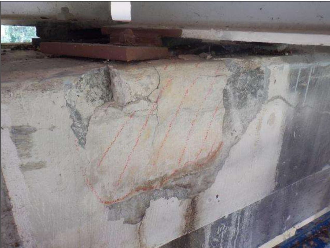
Span 4 Beam 3 - Far Bearing: NEW BEARING HAS A LOSS OF BEARING AREA DUE TO SPALL ON CAP. AREA REPAIRED IS UNSOUND AND HAS 6 IN HIGH X 5 IN WIDE X 2 IN DEEP SPALLS. (PAR)
