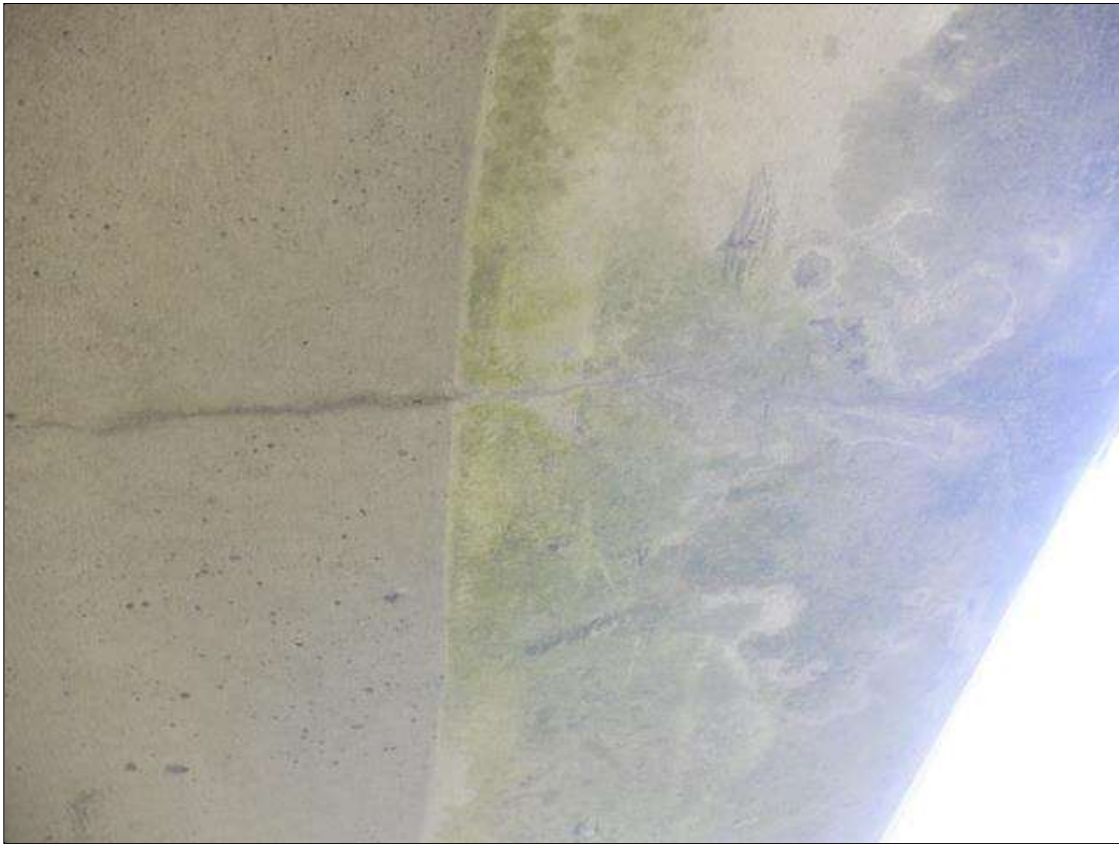
Span 8 Deck: UP TO .05 IN WIDE X 3 FT LONG HORIZONTAL CRACKS UNDER RIGHT OVERHANG SIMILAR UNDER LEFT OVERHANG
