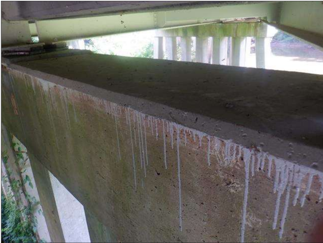
TYPICAL PAINT ON BENT 1, BAY 3. TYPICAL IN ALL BAYS
