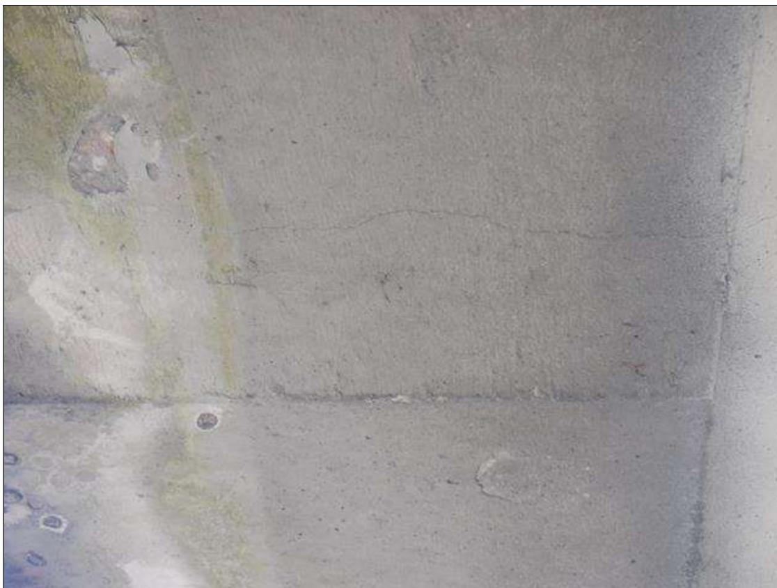
Span 4 Deck: EIGHT (8) UP TO 0.02 IN WIDE X UP TO 3 FT LONG TRANSVERSE CRACKS IN LEFT OVERHANG.
