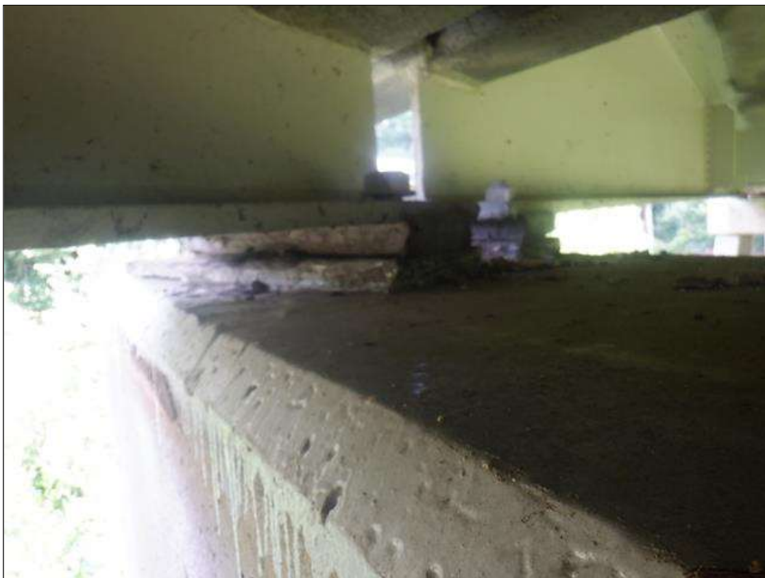
Span 1 Far Bearing: BEARINGS HAVE BEEN PAINTED SINCE PREVIOUS INSPECTION. SECTION LOSS EXISTS BENEATH THE PAINTED SURFACES IN BOTH MASONRY AND SOLE PLATES. UP TO 85% SECTION REMAINING.
