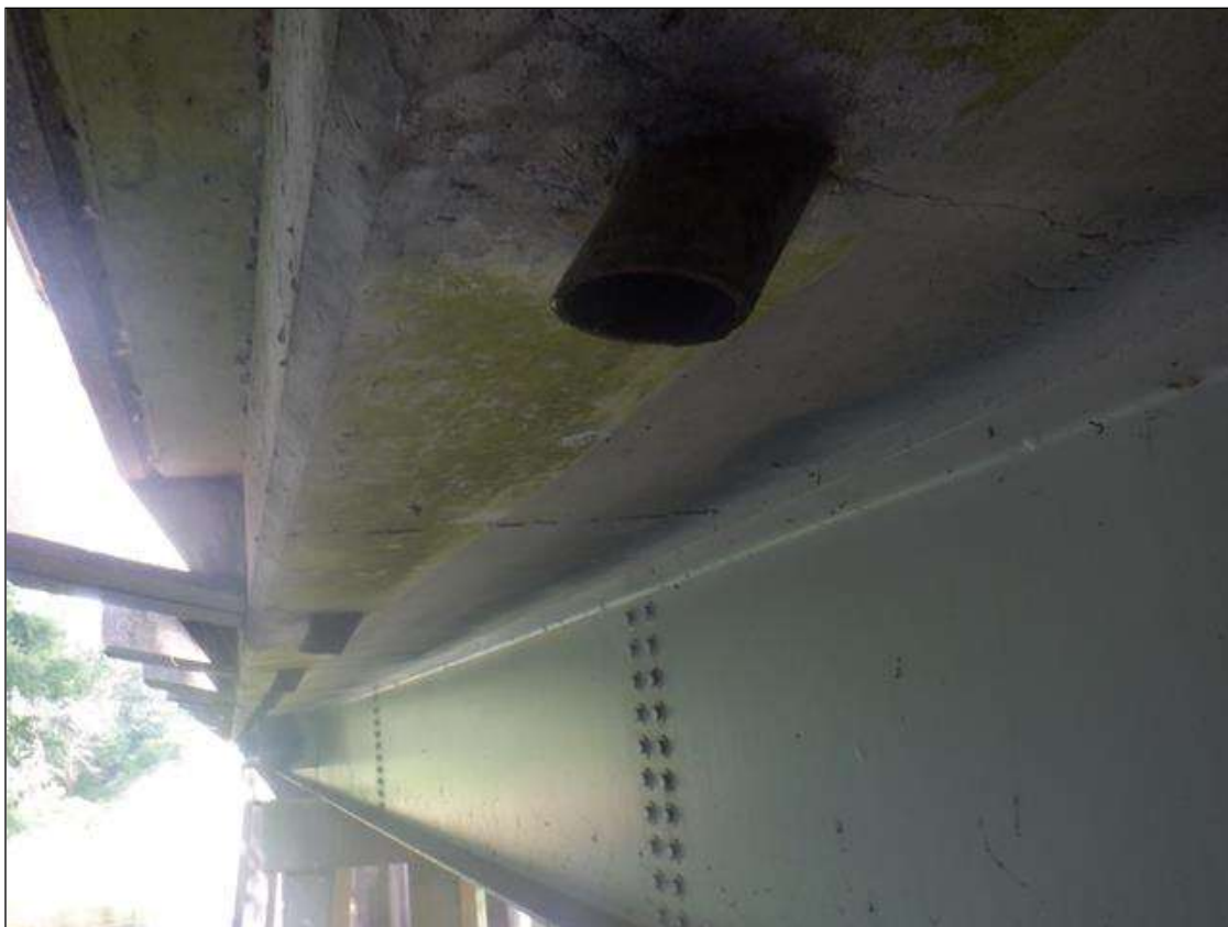
TYPICAL DRAINAGE PIPES UNDER RIGHT OVERHANG IN SPAN 8. SIMILAR IN ALL SPANS AND UNDER LEFT OVERHANG
