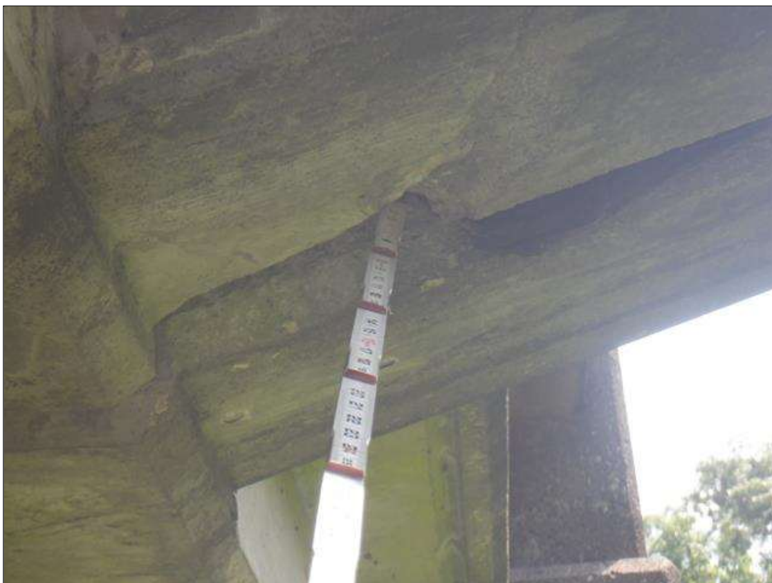
Span 1 Deck: 9 IN LONG X UP TO 4 IN WIDE X UP TO 2.5 IN DEEP SPALL IN RIGHT DECK OVERHANG ABOVE BENT 1.
