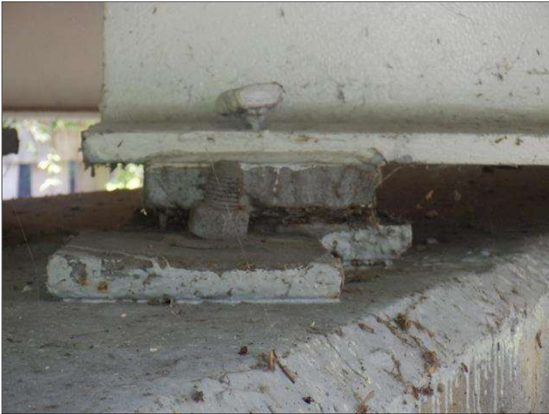
Span 8 Near Bearing: BEARINGS HAVE BEEN PAINTED SINCE PREVIOUS INSPECTION. SECTION LOSS EXSISTS BENEATH THE PAINTED SURFACES IN BOTH MASONRY AND SOLE PLATES. UP TO 95% SECTION REMAINING.
