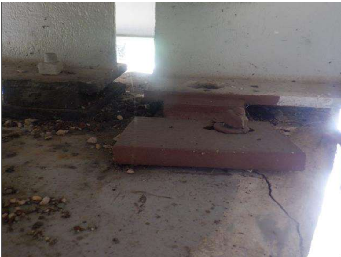
Span 4 Beam 3 - Far Bearing: BEARING HAS WELDED REPAIR WITH NEW ANCHOR BOLTS.
