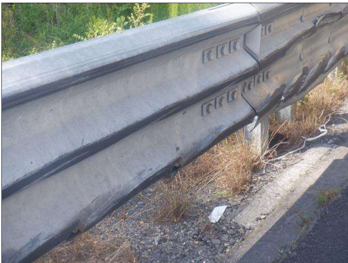
HEAVY IMPACT DAMAGE FOR 10 FT LONG IN SOUTHEAST APPROACH GUARDRAIL AT 15 FT FROM END BENT 1
