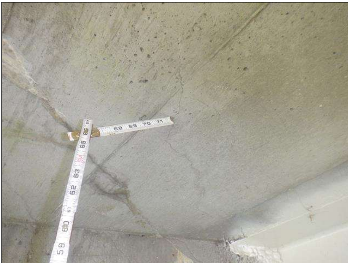
Span 1 Deck: UP TO 0.02 IN WIDE TRANSVERSE CRACKS IN DECK UNDERSIDE IN BAY 1 BETWEEN INTERMEDIATE DIAPHRAGMS TYPICAL IN BAYS 2 AND 3.
