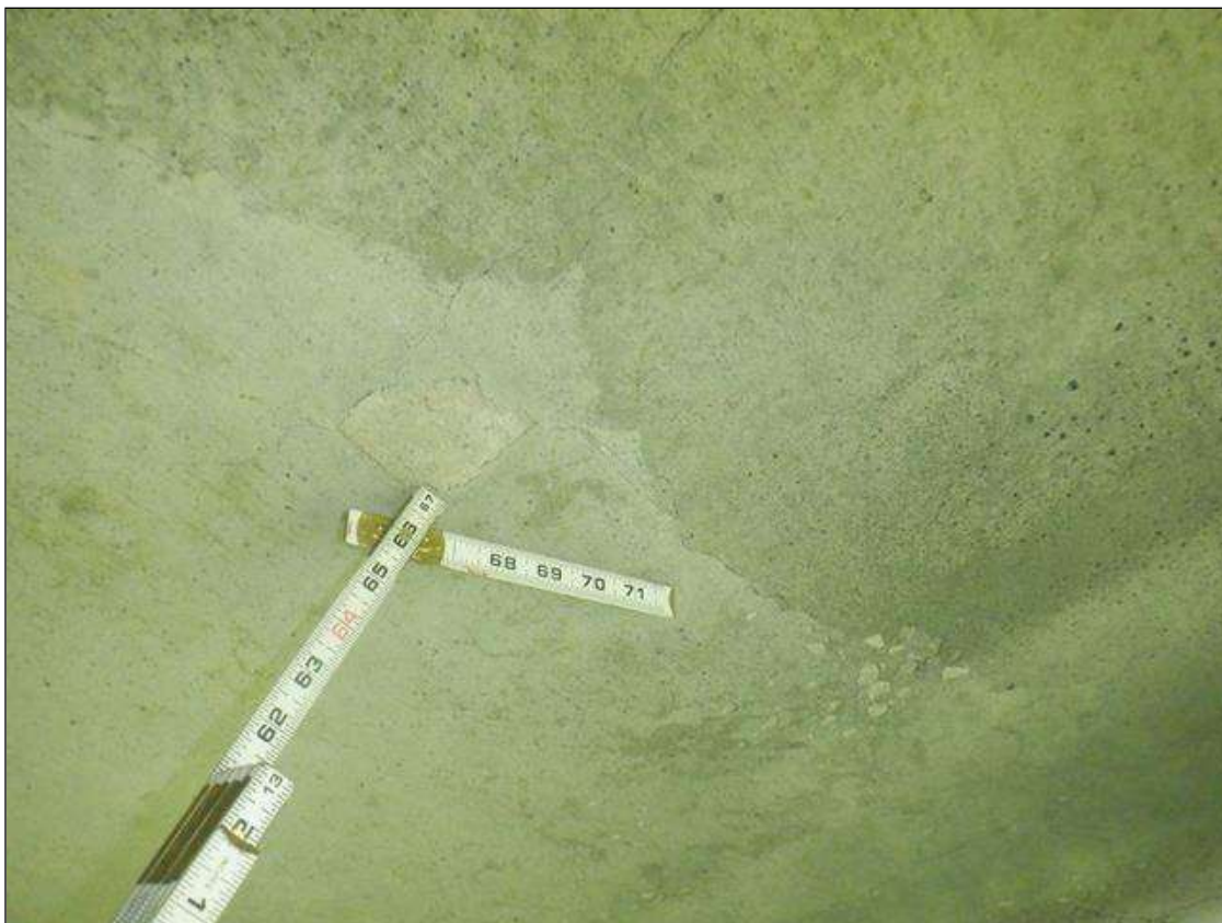
Span 2 Deck: UP TO 0.02 IN WIDE RANDOM CRACKING IN DECK UNDERSIDE, SCATTERED THROUGHOUT.
