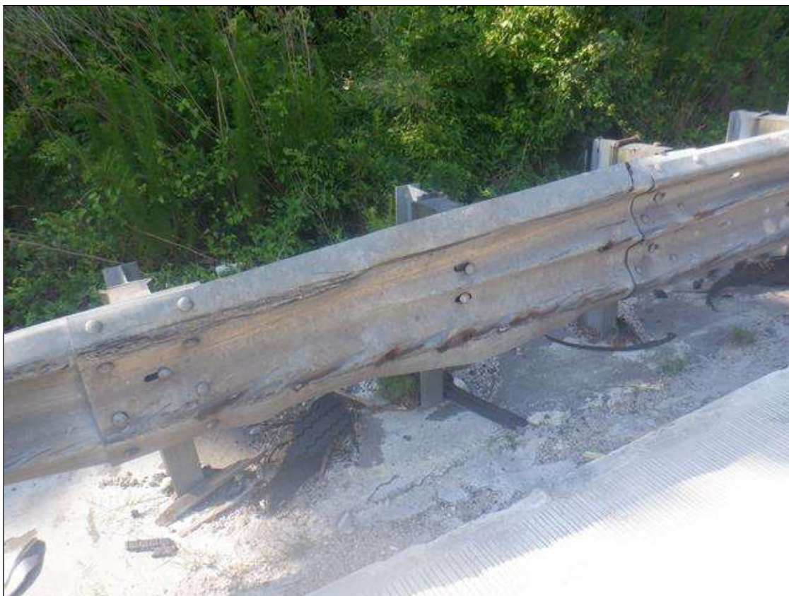
MODERATE IMPACT DAMAGE TO NORTHEAST APPROACH GUARDRAIL AT 15 FT FROM END BENT 2
