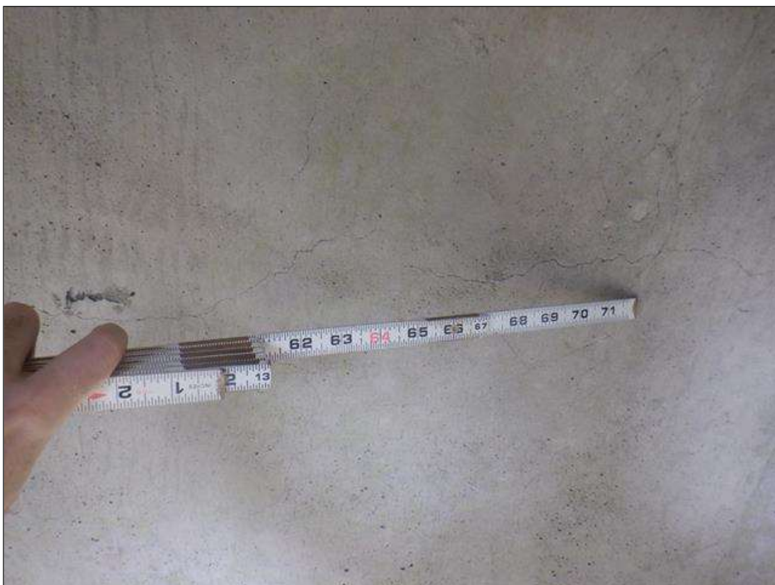
Span 4 Deck: UP TO 0.02 IN WIDE RANDOM CRACKING IN DECK UNDERSIDE, SCATTERED THROUGHOUT.
