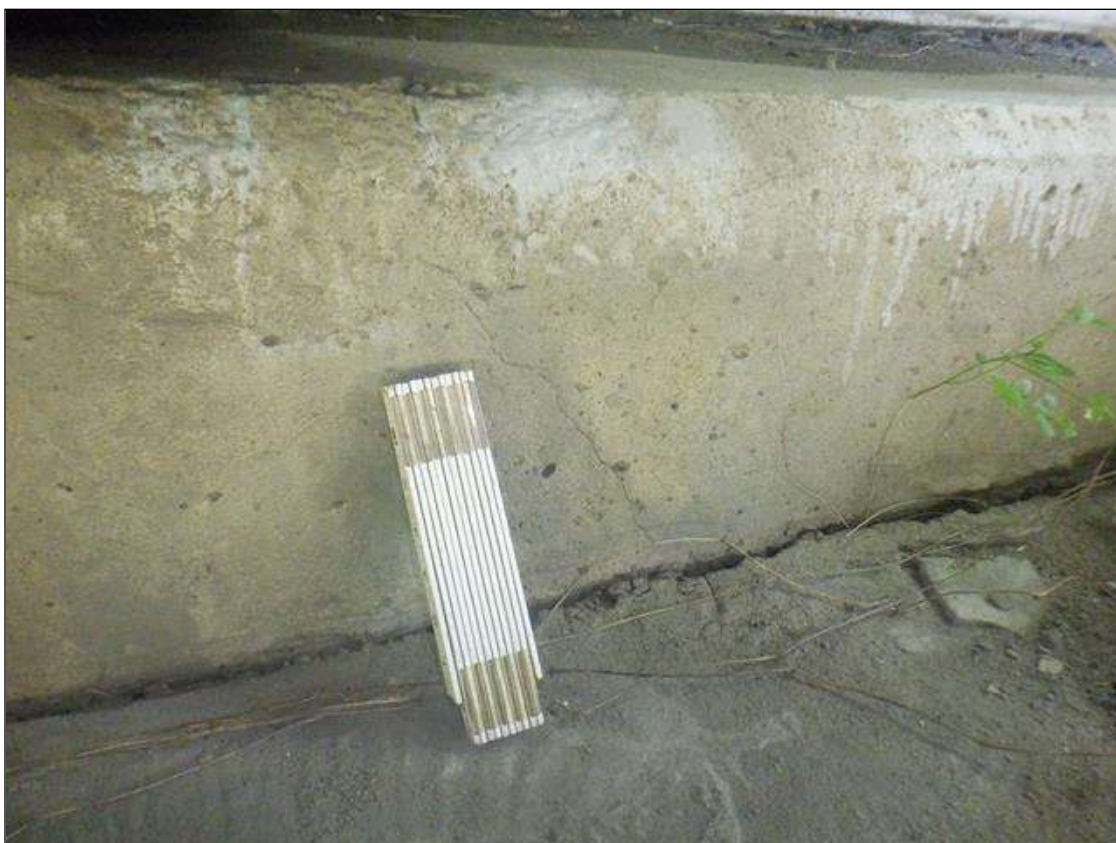
End Bent 2 Cap 1: 2 FT HIGH X 1/16 IN WIDE DIAGONAL CRACK UNDER BEAM 4.
