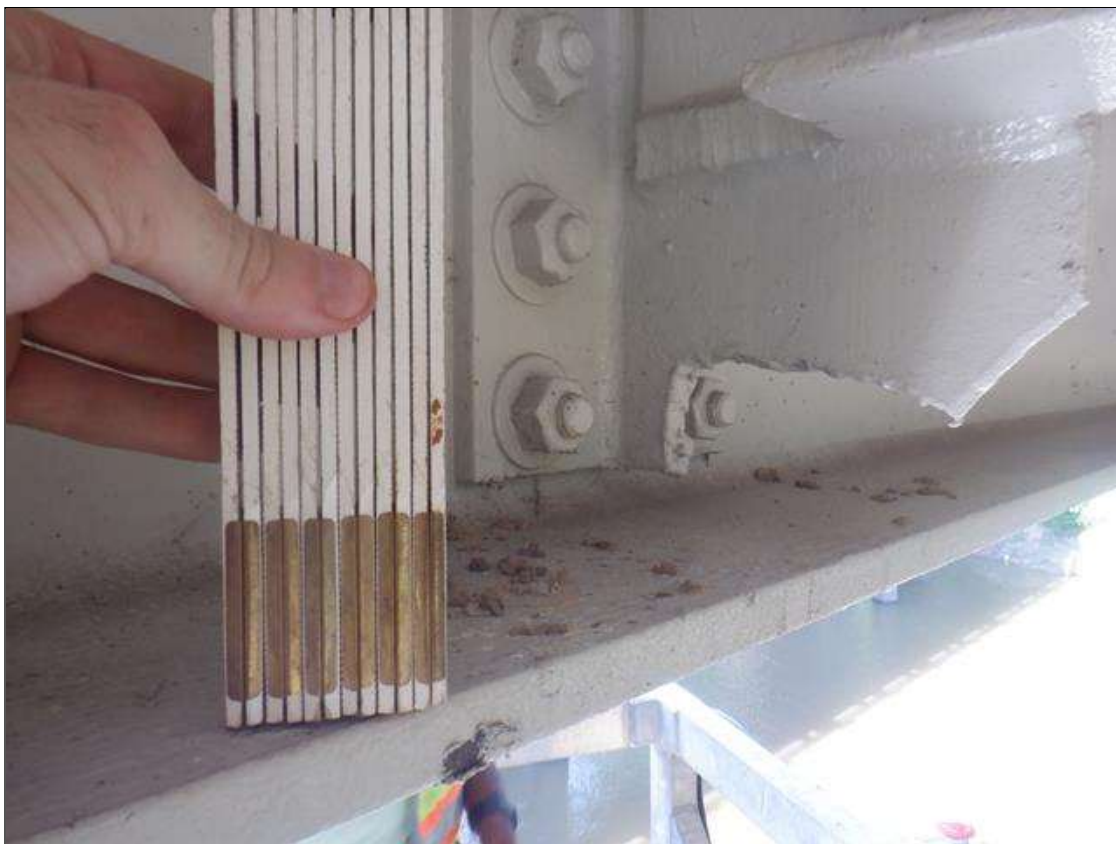
Span 4 Beam 1: 2 IN HIGH OF INTERMEDIATE STIFFENER IS CUT OUT AT BOTH LOCATIONS. PAR IS NOT ISSUED AS IT APPEARS TO BE FROM PREVIOUS BRIDGE REPAIR.
