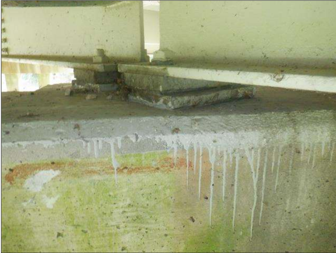
Span 2 Far Bearing: BEARINGS HAVE BEEN PAINTED SINCE PREVIOUS INSPECTION. SECTION LOSS EXISTS BENEATH THE PAINTED SURFACES IN BOTH MASONRY AND SOLE PLATES. UP TO 85% SECTION REMAINING.
