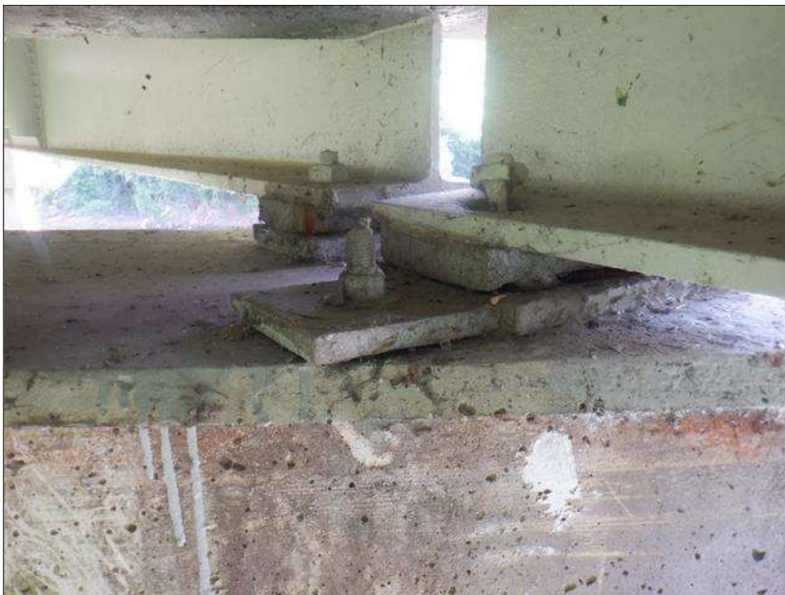
Span 2 Far Bearing: WELDED REPAIR WITH NEW ANCHOR BOLT. UP TO 50% SECTION LOSS IN OLD ANCHOR BOLT. PAR NOT ISSUED DUE TO NEW ANCHOR BOLT REPAIR.
