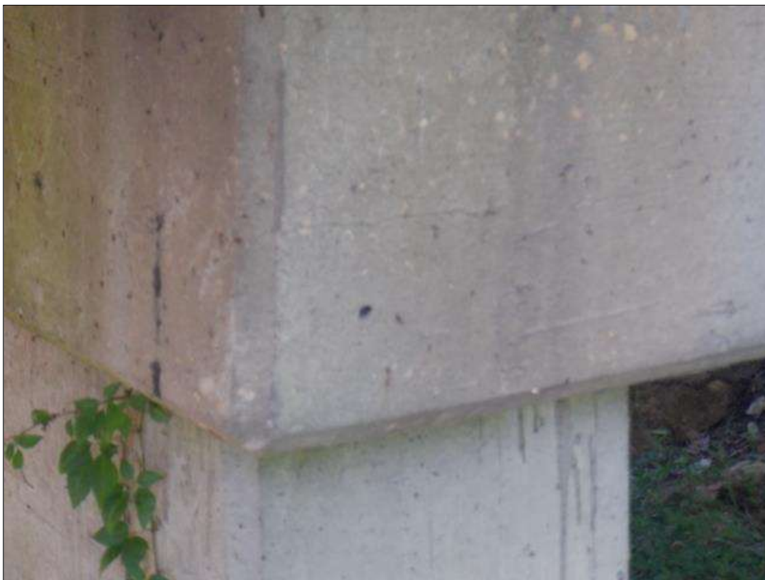
Bent 7 Cap 1: HAIRLINE HORIZONTAL CRACKS IN BOTH ENDS
