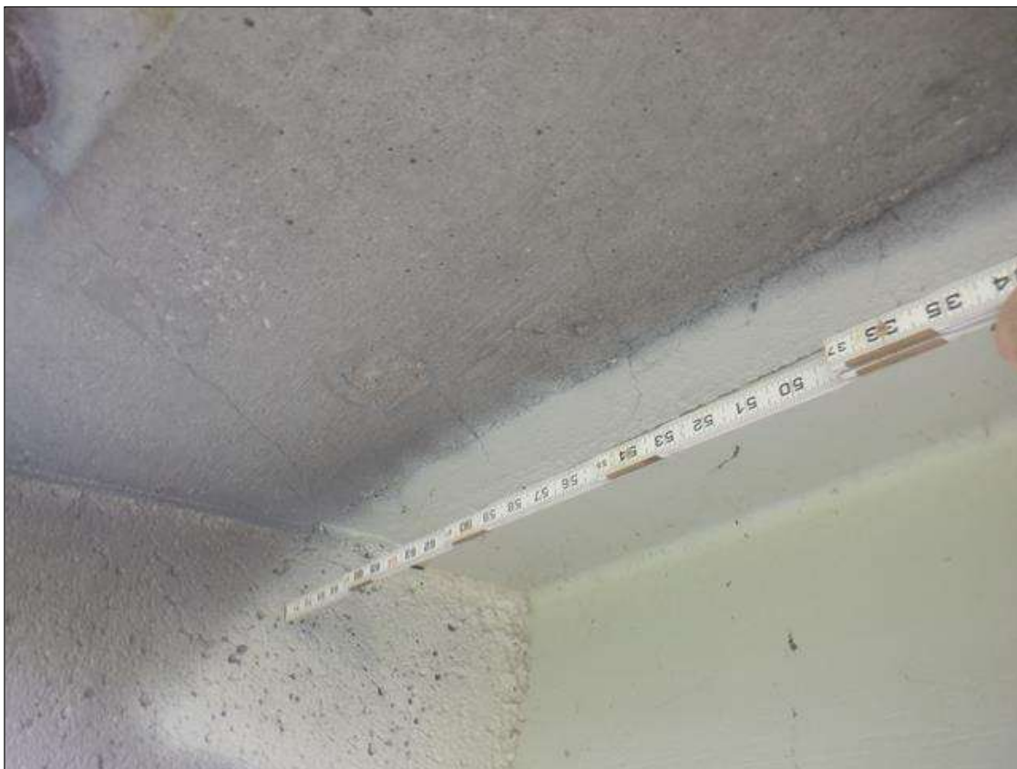
Span 1 Deck: SIX (6) UP TO 0.02 IN WIDE TRANSVERSE CRACKS UNDER LEFT OVERHANG, SCATTERED.
