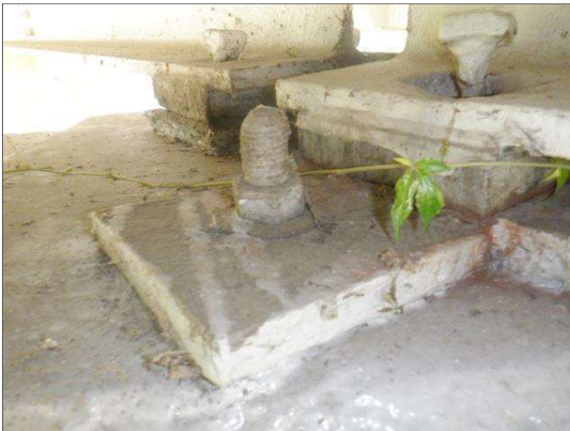
Span 8 Beam 3 - Near Bearing: BEARING ASSEMBLY HAS WELDED REPAIR WITH NEW ANCHOR BOLT.
