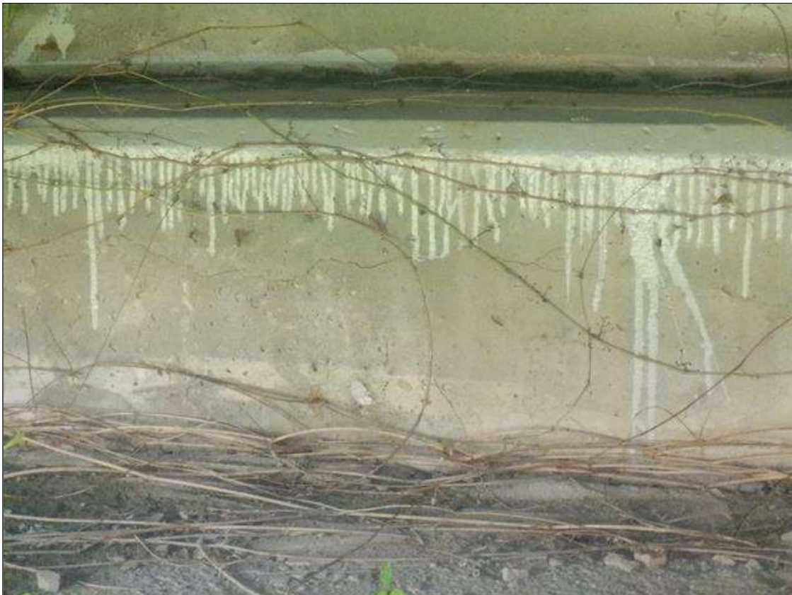
End Bent 2 Cap 1: 3 FT LONG X UP TO 1/16 IN WIDE HORIZONTAL CRACK, BELOW BAY 1.
