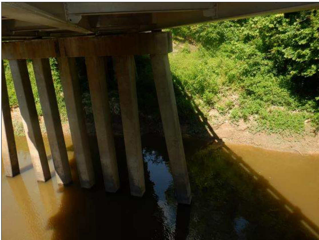
50 FT LONG X 4 FT HIGH X 4 FT DEEP AREA OF EROSION ALONG NORTH BANK
