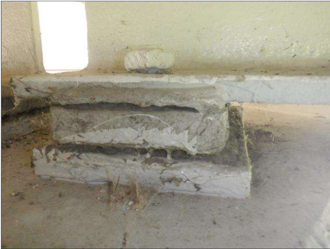
Span 3 Far Bearing: BEARINGS HAVE BEEN PAINTED SINCE PREVIOUS INSPECTION. SECTION LOSS EXISTS BENEATH THE PAINTED SURFACES IN BOTH MASONRY AND SOLE PLATES. UP TO 80% SECTION REMAINING.
