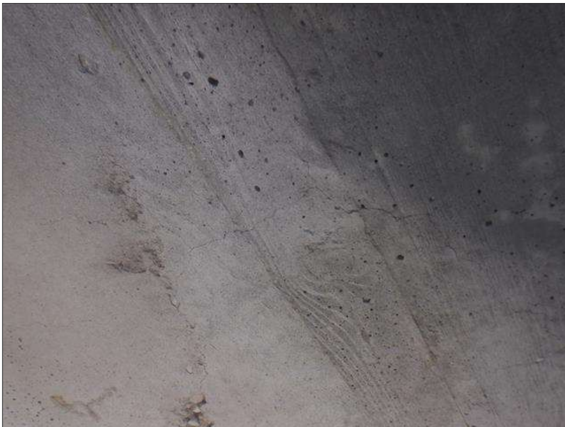
Span 6 Deck: UP TO 0.02 IN WIDE RANDOM CRACKING IN DECK UNDERSIDE, SCATTERED THROUGHOUT.
