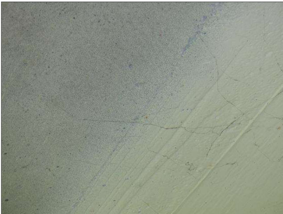
Span 3 Deck: SIX (6) UP TO 0.02 IN WIDE X UP TO 3 FT LONG TRANSVERSE CRACKS IN RIGHT OVERHANG. TYPICAL AT LEFT OVERHANG.
