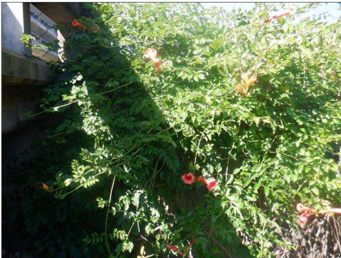
HEAVY VEGETATION GROWTH AT SOUTHWEST, SOUTHEAST, AND NORTHWEST WINGWALL
