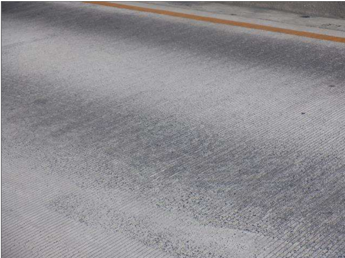
Span 1 Wearing Surface: MINOR ABRASION WITH EXPOSED AGGREGATE ALONG THE WHEEL PATHS FOR FULL LENGTH
