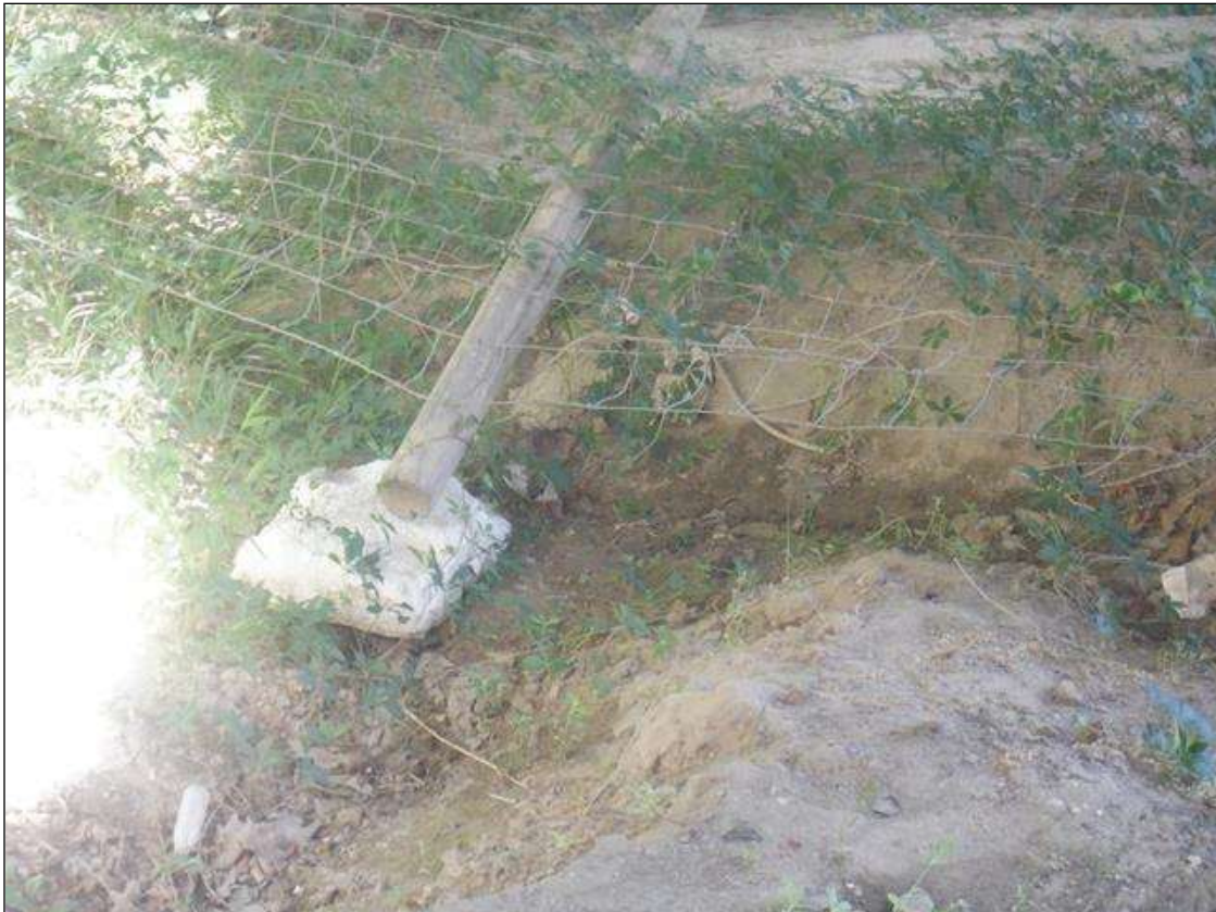
5 FT LONG X 20 FT WIDE AREA OF EROSION WITH FALLEN FENCE POST UNDER SPAN 8
