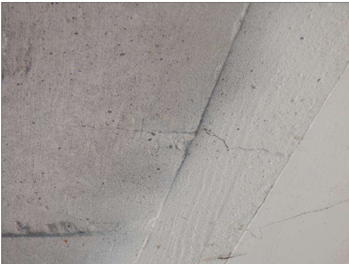
Span 6 Deck: FOUR (4) UP TO 0.02 IN WIDE X UP TO 3 FT LONG TRANSVERSE CRACKS IN RIGHT OVERHANG. SEVEN (7) SIMILAR CRACKS IN LEFT OVERHANG.
