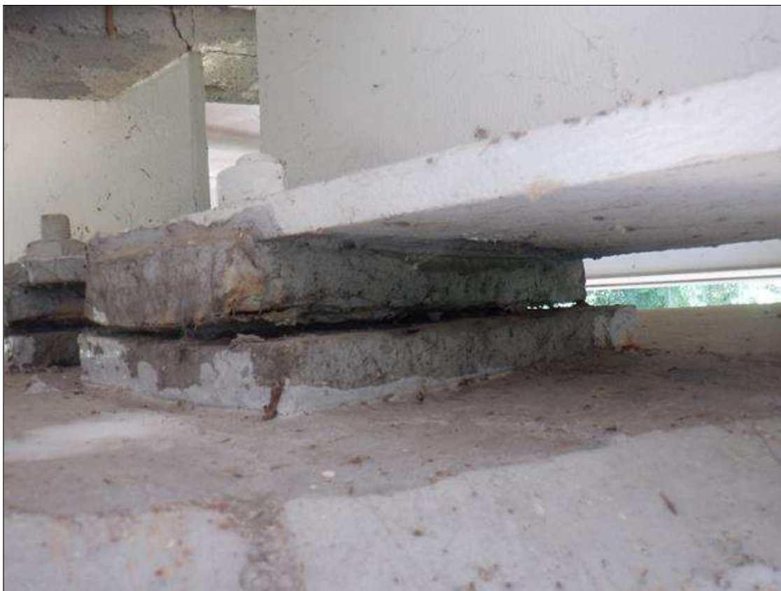
Span 5 Far Bearing: BEARINGS HAVE BEEN PAINTED SINCE PREVIOUS INSPECTION. SECTION LOSS EXISTS BENEATH THE PAINTED SURFACES IN BOTH MASONRY AND SOLE PLATES. UP TO 95% SECTION REMAINING.
