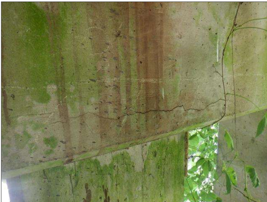
Bent 7 Cap 1: 3 FT WIDE X 6 IN HIGH DELAMINATION WITH A 3 FT LONG HORIZONTAL CRACK UP TO 1/32 IN WIDE BOTTOM OF NORTH FACE, OVER PILE 3.
