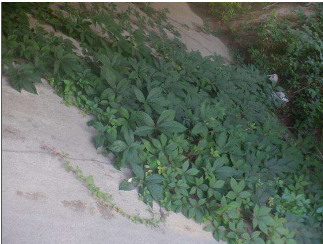
HEAVY VEGETATION GROWTH FOR FULL HEIGHT OF SLOPE PROTECTION AT END BENT 2 UNDER BAY 1
