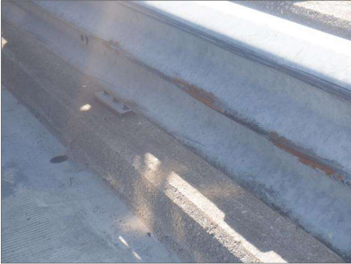
Span 1 Right Bridge Rail: IMPACT DAMAGE WITH SCRAPE MARKS FOR FULL SPAN LENTH IN BOTTOM OF SUPPLEMENTAL RAIL.
