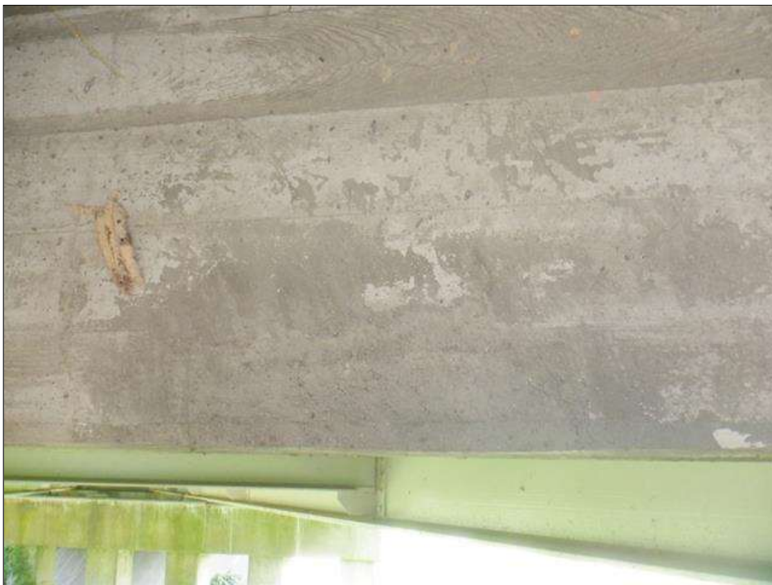
Span 3 Deck: 2 FT LONG X 1 FT HIGH SOUND CONCRETE PATCH IN BAY 2 BENT DIAPHRAGM AT BENT 2
