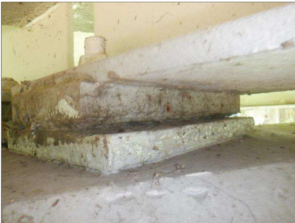
Span 3 Near Bearing: BEARINGS HAVE BEEN PAINTED SINCE PREVIOUS INSPECTION. SECTION LOSS EXSISTS BENEATH THE PAINTED SURFACES IN BOTH MASONRY AND SOLE PLATES. UP TO 95% SECTION REMAINING.
