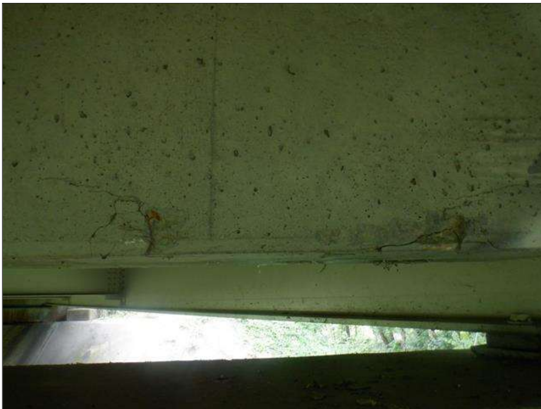
Span 2 Deck: TWO (2) AREAS OF UNSOUND CONCRETE UP TO 2.5 FT LONG X 1 FT HIGH WITH SPALLING UP TO 5 IN DIAMETER X UP TO 1 IN DEEP IN END DIAPHRAGM IN BAY 1 AT BENT 1.
