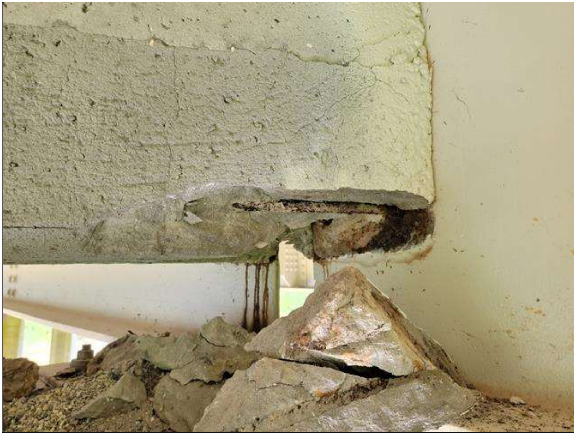
Span 7 Deck: 1 FT LONG X 6 IN HIGH X 12 IN WIDE SPALL WITH EXPOSED REBAR IN BAY 3 END DIAPHRAGM AT BENT 6. 90% SECTION REMAINING IN THE EXPOSED REBAR.
