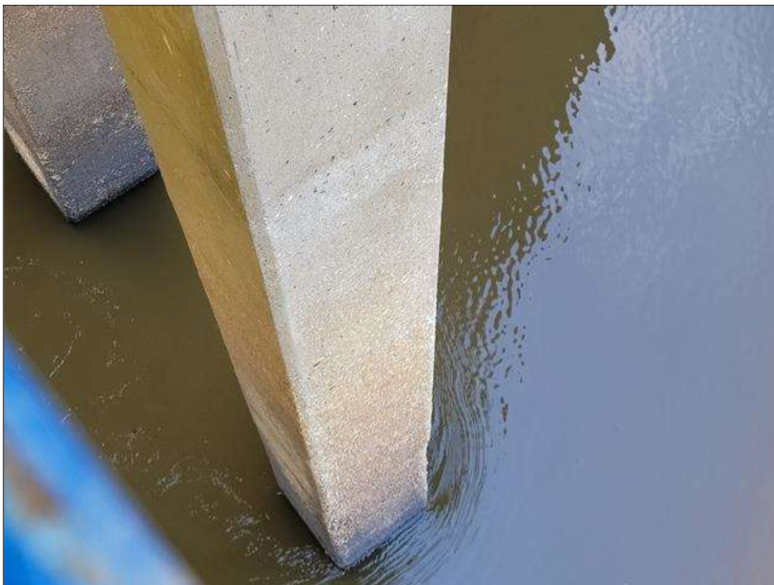
Bent 5 Pile 1: ABRASION WITH COARSE AGGREGATE EXPOSED 1/16 IN TO 1/4 IN LOSS OF FACIAL CONCRETE IN UPSTREAM FACE.
