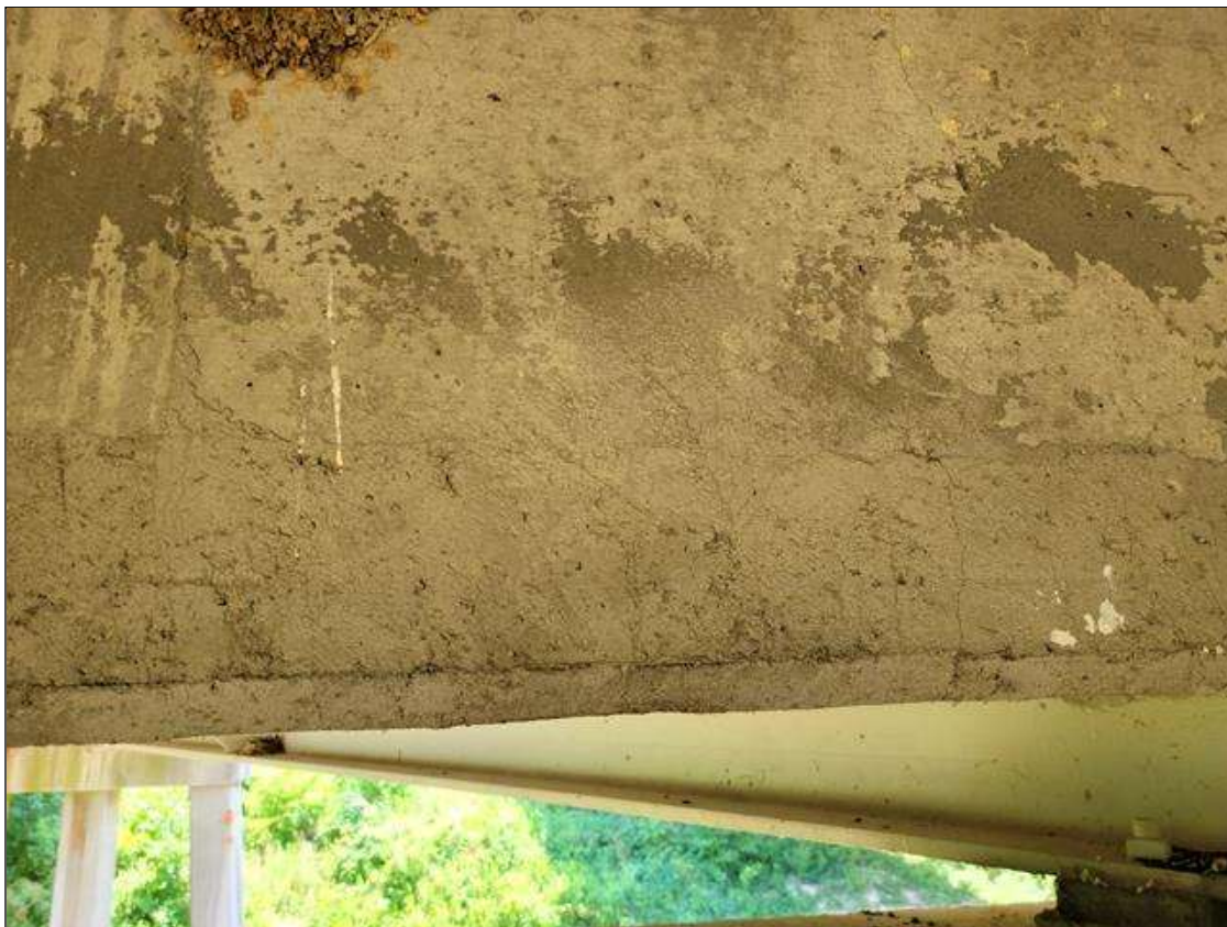
Span 5 Deck: 8 FT LONG X 6 IN HIGH UNSOUND CONCRETE PATCH WITH HAIRLINE CRACKS IN BAY 2 END DIAPHRAGM, AT BENT 5.
