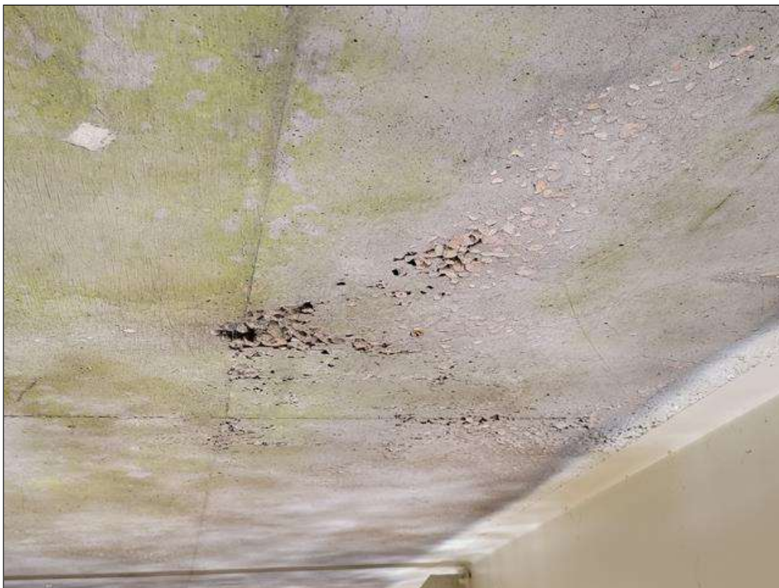
Span 5 Deck: 6 FT LONG X 3 FT WIDE X UP TO 3/4 IN DEEP AREA OF HONEYCOMBING IN BAY 3 NEAR BENT 5.
