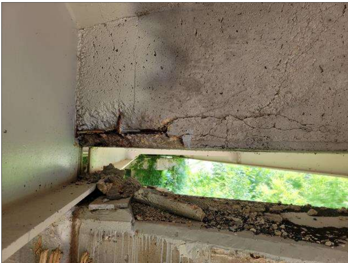
Span 6 Deck: 2.5 FT WIDE X 10 IN LONG X UP TO 6 IN HIGH AREA OF UNSOUND CONCRETE AND SPALL UP TO 2 IN DEEP WITH EXPOSED REINFORCEMENT IN BAY 3 END DIAPHRAGM AT BENT 6. 90% SECTION REMAINING IN EXPOSED REBAR.
