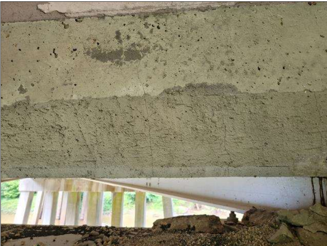
Span 7 Deck: 6 FT LONG X 12 IN HIGH SOUND CONCRETE PATCH BOTTOM OF BAY 3 END DIAPHRAGM, NEXT TO BEAM 3, AT BENT 6. PATCH EXHIBITS UP TO 0.03 IN WIDE VERTICAL CRACKS, SCATTERED.
