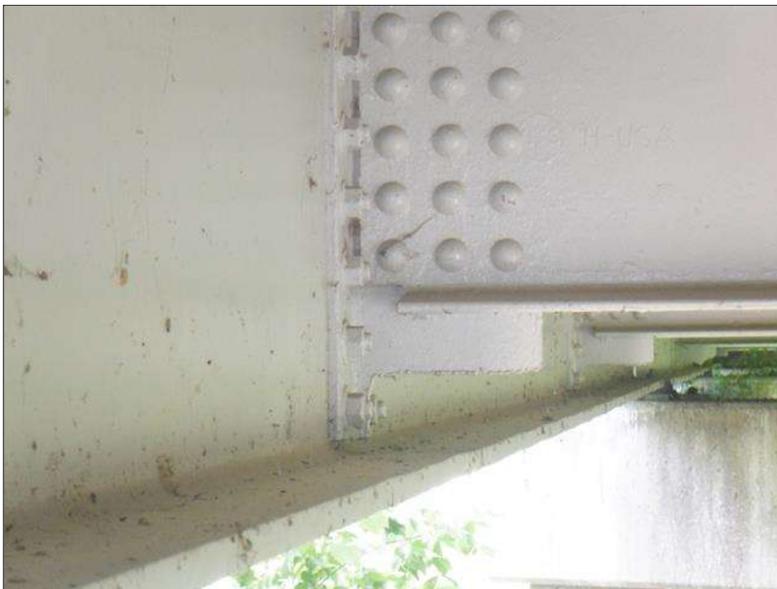
Span 3 Beam 4: UP TO 2 IN HIGH OF SECTION CUT OUT AT BOTTOM OF INTERMEDIATE STIFFENER. PAR IS NOT ISSUED AS IT APPEARS TO BE FROM A BRIDGE REPAIR
