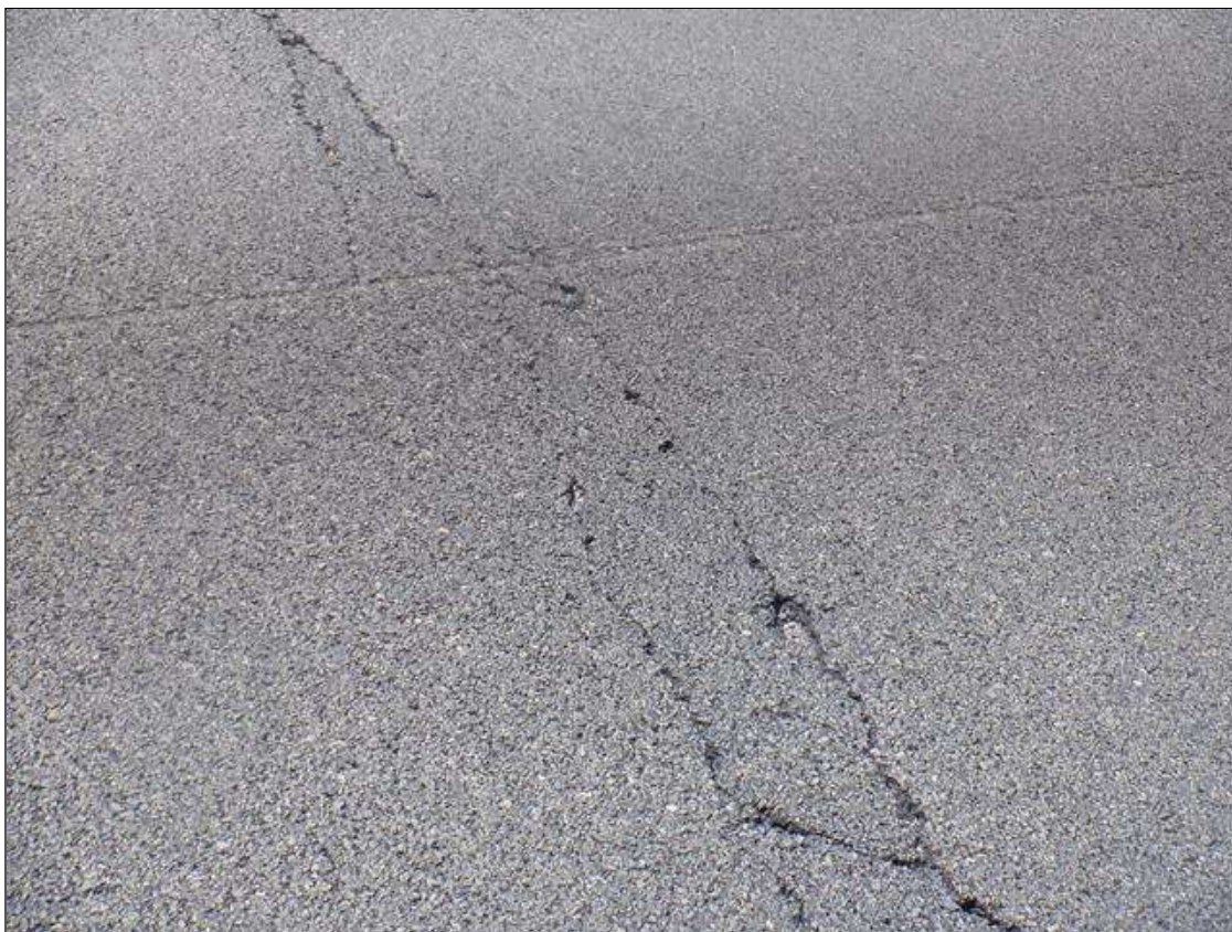
8 IN LONG X FULL TRAVEL LANE WIDTH OF UNSOUND ASPAHLT PAVEMENT IN NORTH APPROACH AT 15 FT FROM END OF APPROACH SLAB
