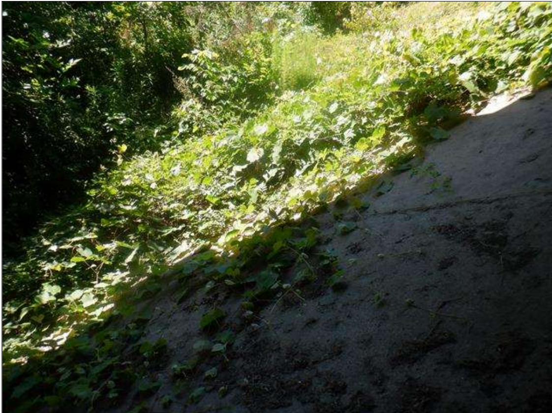
HEAVY VEGETATION GROWTH FOR FULL HEIGHT OF SLOPE PROTECTION AT END BENT 1 UNDER BAY 1
