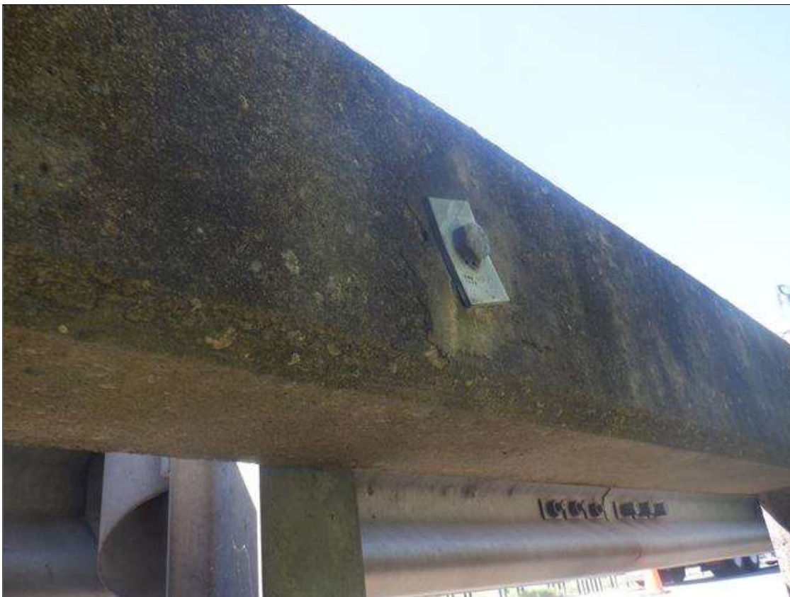
Span 1 Left Bridge Rail: NEW REPAIR: 6 IN DIAMETER SOUND CONCRETE PATCH AT ANCHOR BOLT CONNECTION TO SUPPLEMENTAL GUARDRAIL
