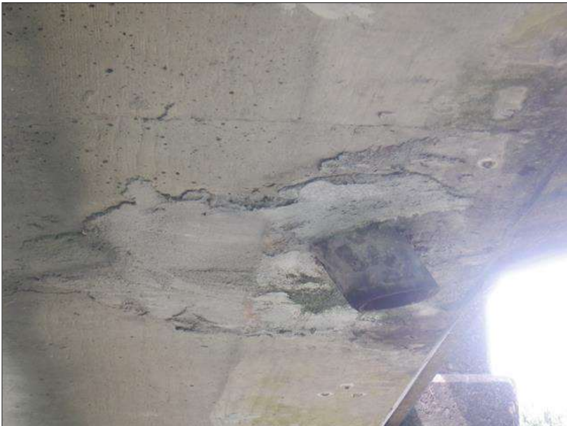
Span 7 Deck: 3 FT X 2 FT AREA OF DELAMINATION, UNDERSIDE OF WEST OVERHANG, AT MID SPAN.
