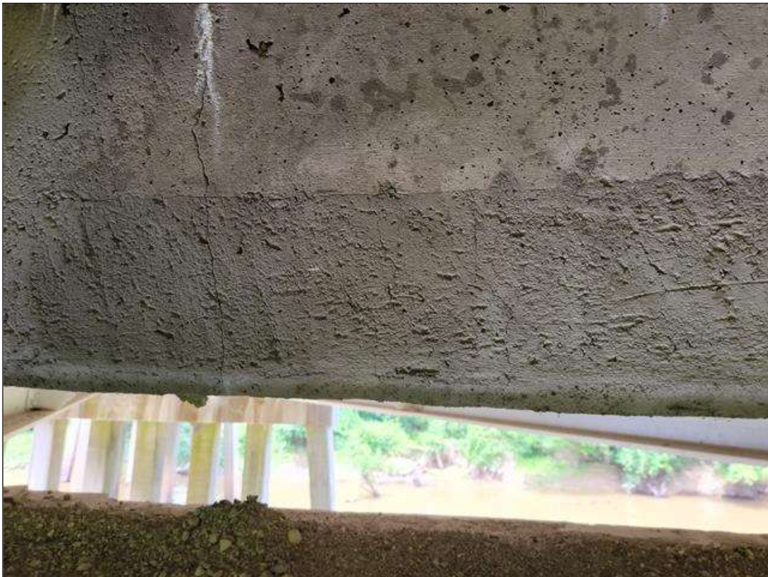
Span 7 Deck: 8 FT LONG X 6 IN HIGH UNSOUND CONCRETE PATCHED AREA WITH UP TO 0.05 IN WIDE VERTICAL AND HORIZONTAL CRACKS IN BAY 2 END DIAPHRAGM, AT BENT 6.
