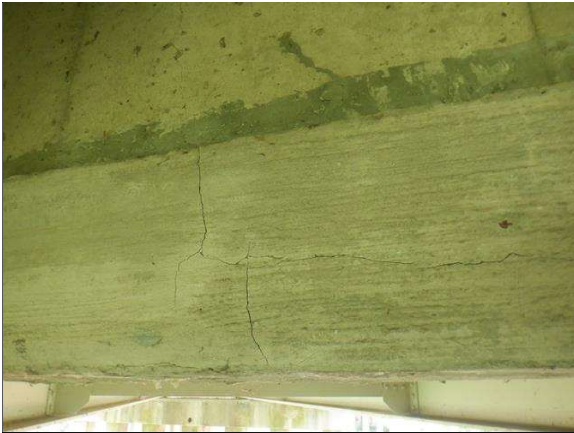
Span 2 Deck: 9 FT LONG X 1 FT HIGH CONCRETE PATCH, BAY 2 END DIAPHRAGM, AT BENT 2. PATCH EXHIBITS UP TO 1/8 IN WIDE X 5 FT LONG CRACK IN THE BOTTOM FACE WITH A 5 FT LONG X 5 IN WIDE UNSOUND CONCRETE AND UP TO 0.02 IN WIDE VERTICAL CRACKS IN FRONT FACE, SCATTERED.
