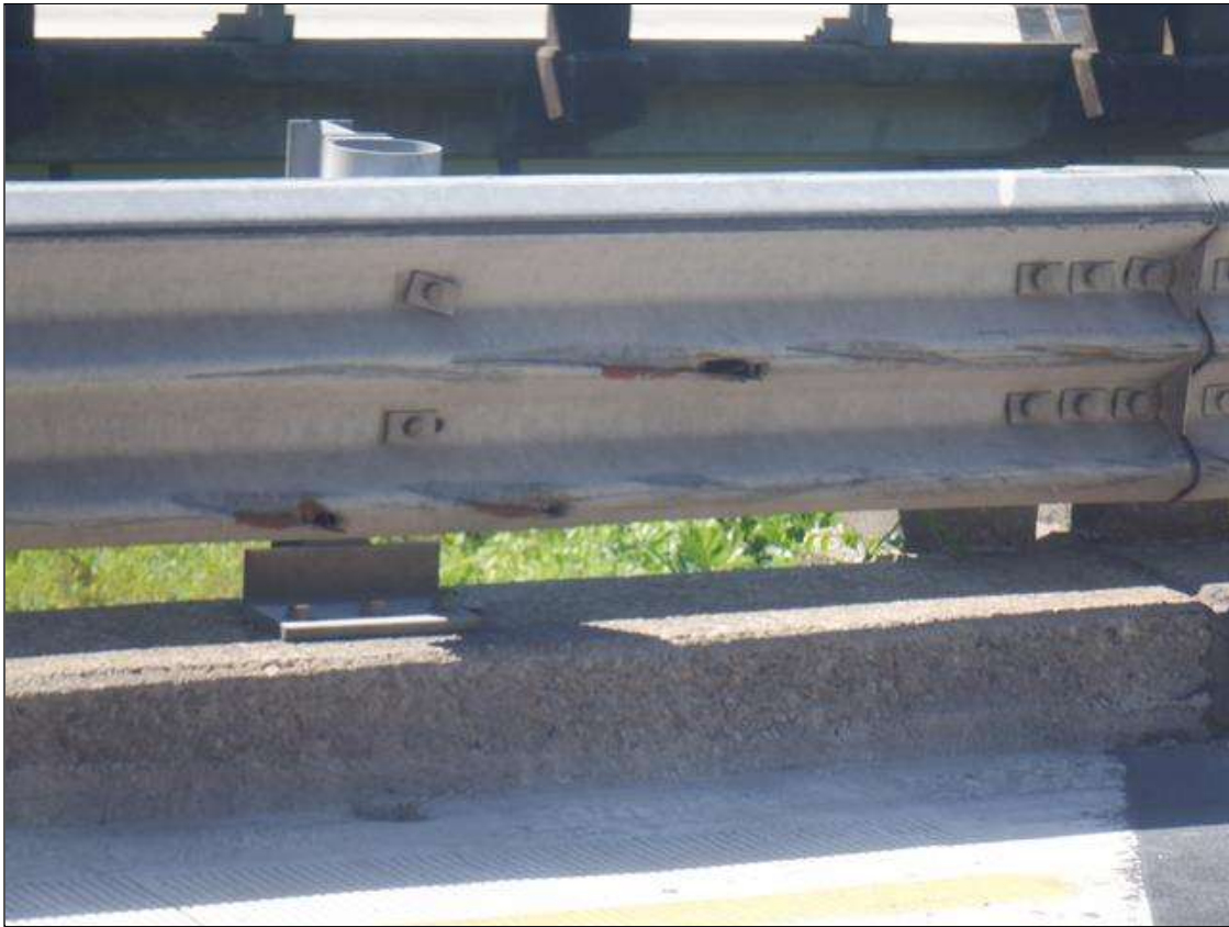
Span 2 Right Bridge Rail: HEAVY IMPACT DAMAGE WITH SCRAPE MARKS AND THROUGH HOLES IN SUPPLEMENTAL GUARDRAIL AT SCATTERED LOCATIONS
