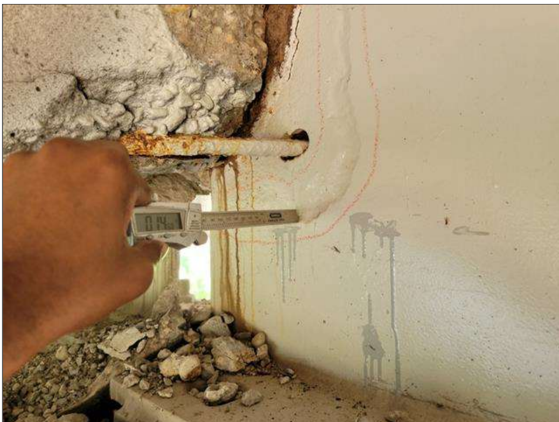
Span 6 Beam 3: UP TO 11 IN HIGH X 10 IN LONG AREA OF SECTION LOSS IN THE WEB BENEATH THE PAINTED SURFACE AT BEAM END AT BENT 6. 0.53 IN SECTION REMAINING.
