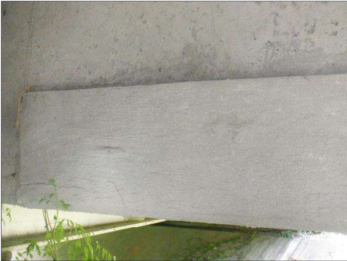
Span 7 Deck: 7 FT LONG X 1 FT HIGH UNSOUND CONCRETE PATCH WITH UP TO 0.05 IN WIDE CRACKS IN INTERMEDIATE DIAPHRAGM IN BAY 3 AT BENT 7.
