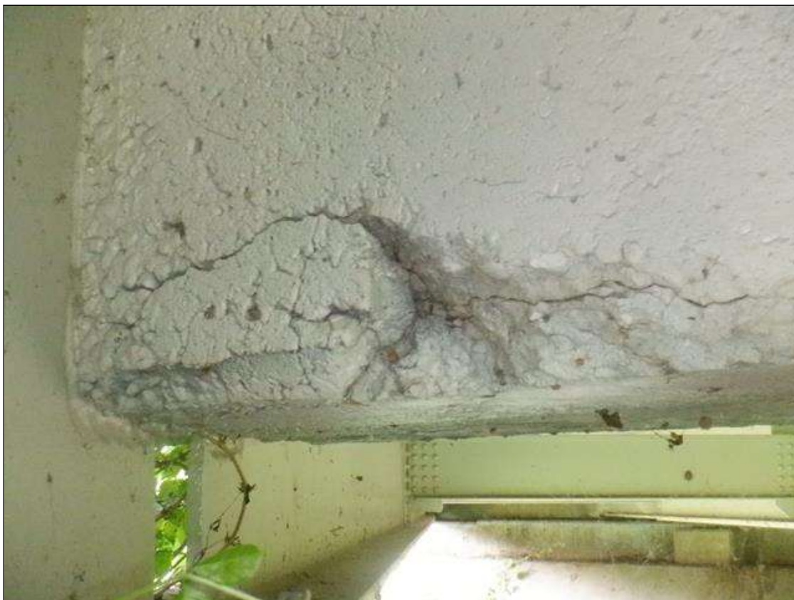
Span 2 Deck: UP TO 1.5 FT WIDE X 4 IN LONG X UP TO 2 IN DEEP SPALL IN DIAPHRAGM IN BAY 3 AT BENT 1.
