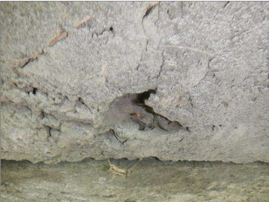
Span 2 Deck: 5 IN DIAMETER X 1 IN DEEP SPALL WITH EXPOSED REINFORCEMENT IN DIAPHRAGM IN BAY 3 AT BENT 1. 90% SECTION REMAINING IN EXPOSED REINFORCEMENT.
