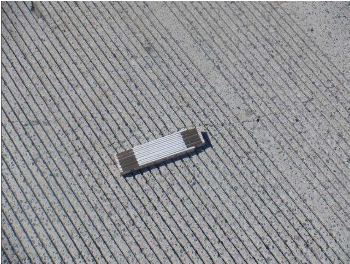
Span 1 Wearing Surface: UP TO 5 FT LONG X 1/16 IN WIDE LONGITUDINAL AND DIAGONAL CRACKS IN BOTH TRAVEL LANES, SCATTERED.
