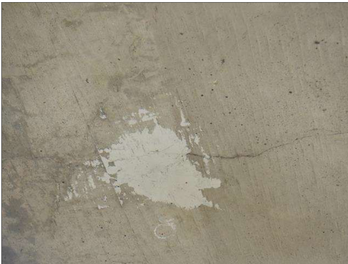
Span 4 Deck: SIX (6) UP TO 0.03 IN WIDE X UP TO 3 FT LONG TRANSVERSE CRACKS IN LEFT OVERHANG.
