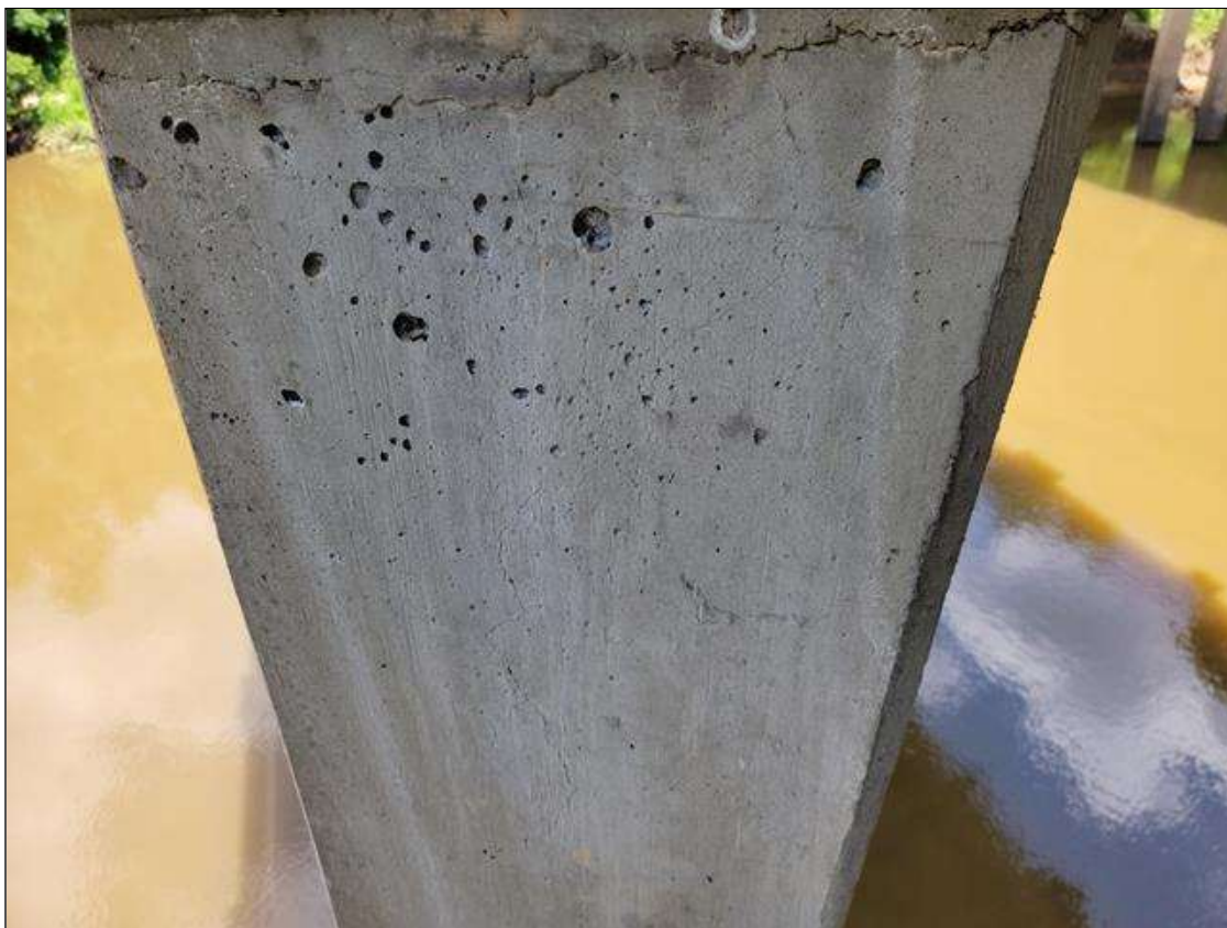
Bent 4 Pile 2: 1 FT LONG VERTICAL HAIRLINE CRACK, SOUTH FACE, BEGINNING AT CAP.
