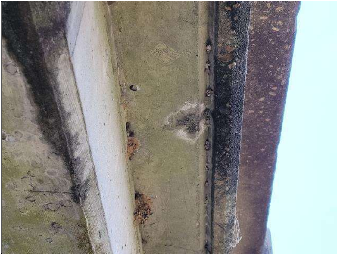
Span 5 Deck: 3 FT LONG X 11 IN HIGH UNSOUND CONCRETE PATCH WITH 1/16 IN WIDE HORIZONTAL CRACK, BAY 2 END DIAPHRAGM, NEXT TO BEAM 2, AT BENT 4.
