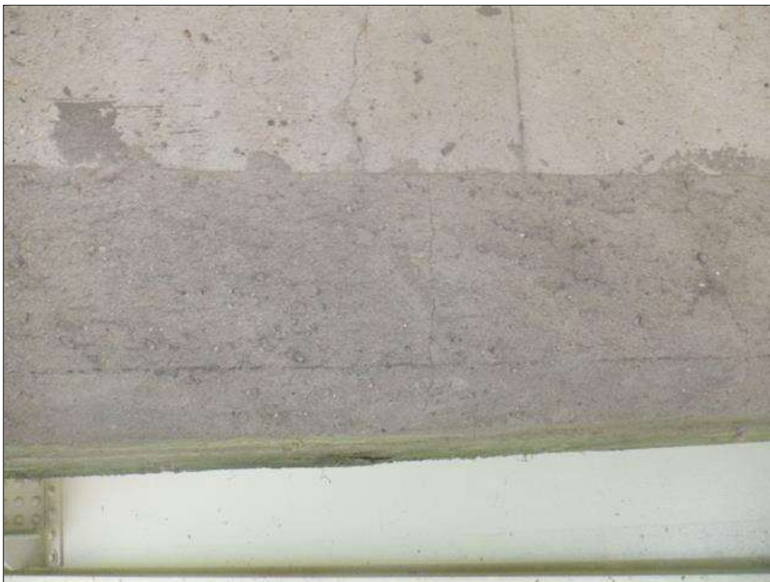
Span 4 Deck: 4 FT LONG X 6 IN HIGH UNSOUND CONCRETE PATCH WITH HAIRLINE VERTICAL CRACKS IN BAY
