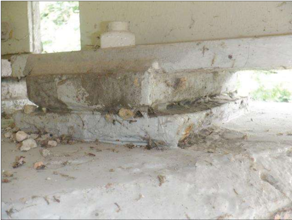
Span 4 Near Bearing: BEARINGS HAVE BEEN PAINTED SINCE PREVIOUS INSPECTION. SECTION LOSS REMAINS BENEATH THE PAINTED SURFACES. UP TO 90% SECTION REMAINING IN BOTH MASONRY AND SOLE PLATES.
