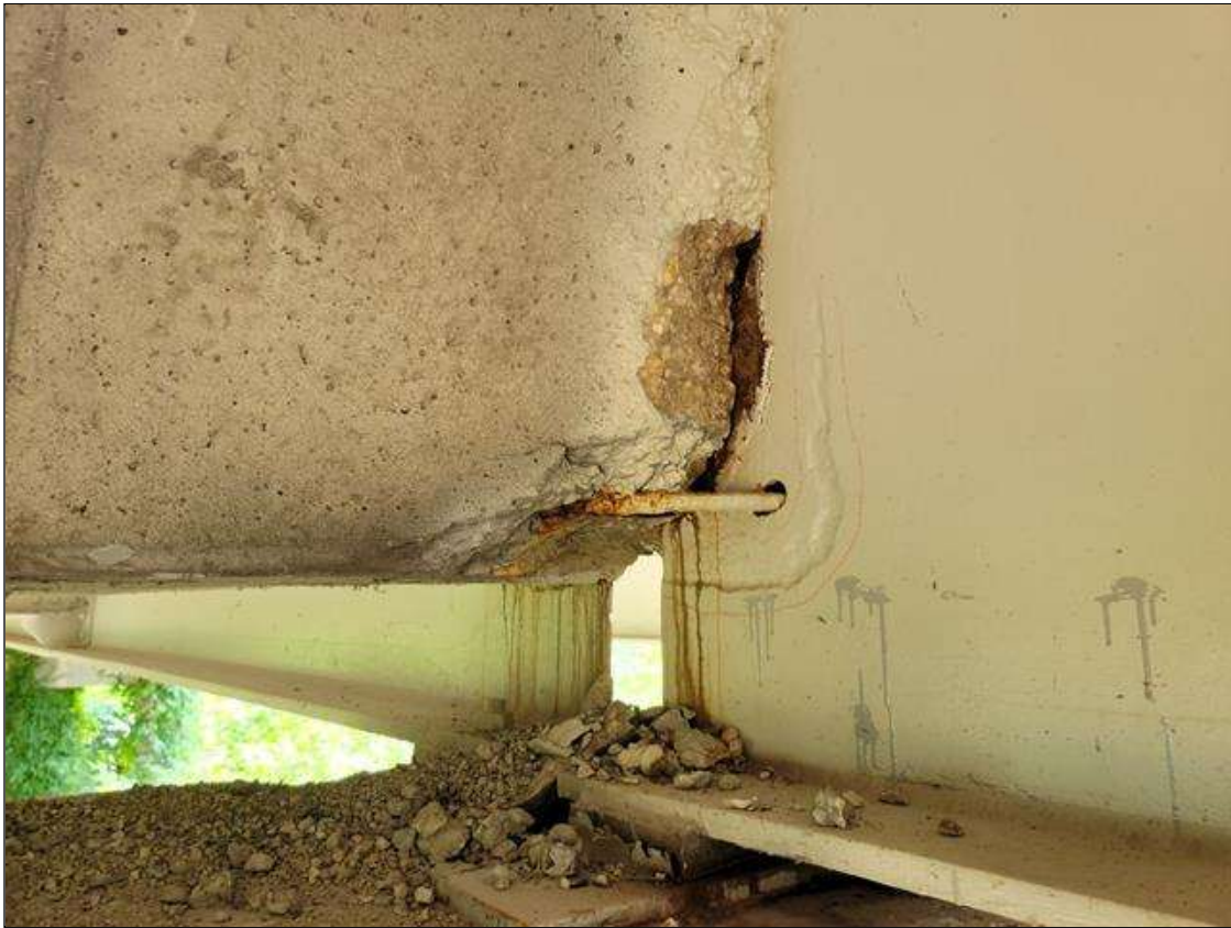
Span 6 Deck: 12 IN WIDE X 9 IN LONG X 14 IN HIGH IN SOUTH FACE SPALL UP TO 3.5 IN DEEP WITH EXPOSED REINFORCEMENT IN BAY 2 AT BENT 6. 90% SECTION REMAINING IN EXPOSED REINFORCEMENT.
