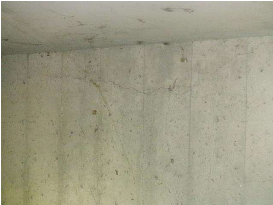
End Bent 1 Abutment: UP 1/16 IN WIDE HORIZONTAL CRACKS AT TOP IN BAYS 2 AND 3
