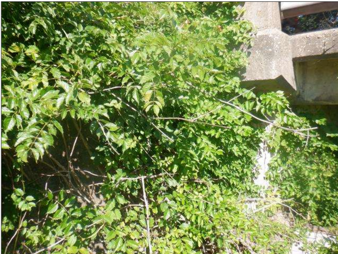
HEAVY VEGETATION GROWTH AT SOUTHEAST AND NORTHWEST WINGWALL
