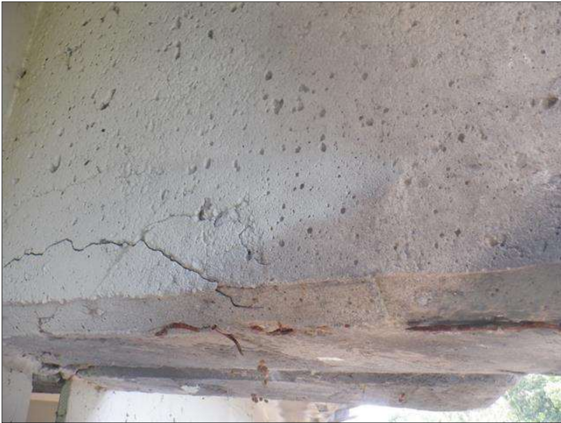
Span 3 Deck: 4 IN HIGH X 1 FT LONG AREA OF UNSOUND CONCRETE WITH 1/8 IN WIDE CRACKS AND EXPOSED REBAR IN END DIAPHRAGM AT BENT 3 UNDER RIGHT OVERHANG. NO MEASURABLE SECTION LOSS IN EXPOSED REBAR.
