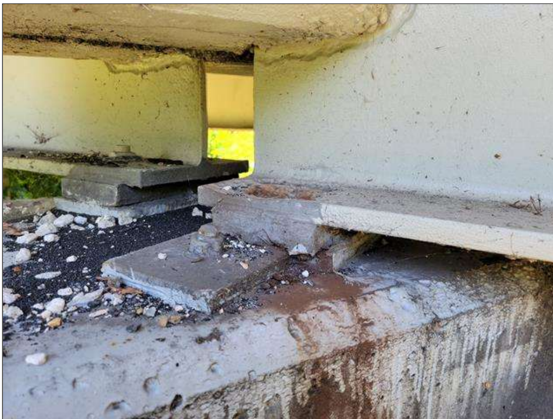
Span 6 Far Bearing: BEARING ASSEMBLY HAS WELDED REPAIR WITH NEW ANCHOR BOLT.
