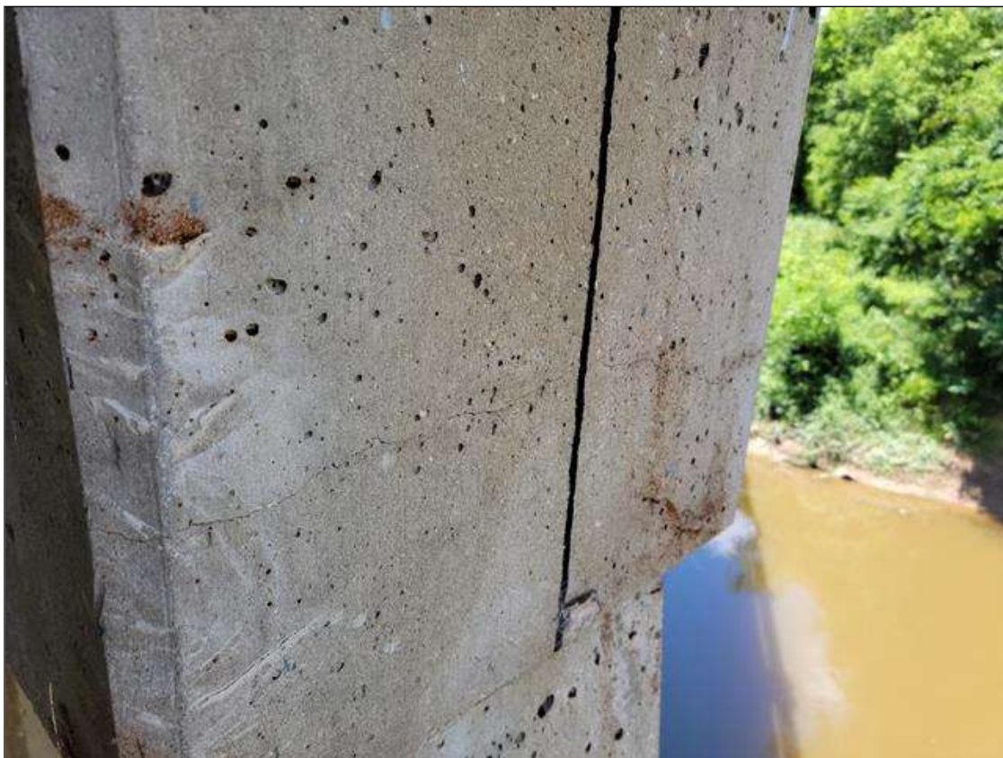
Bent 4 Pile 1: 5 FT LONG X 0.02 IN WIDE VERTICAL CRACK, SOUTH FACE BEGINNING AT CAP.
