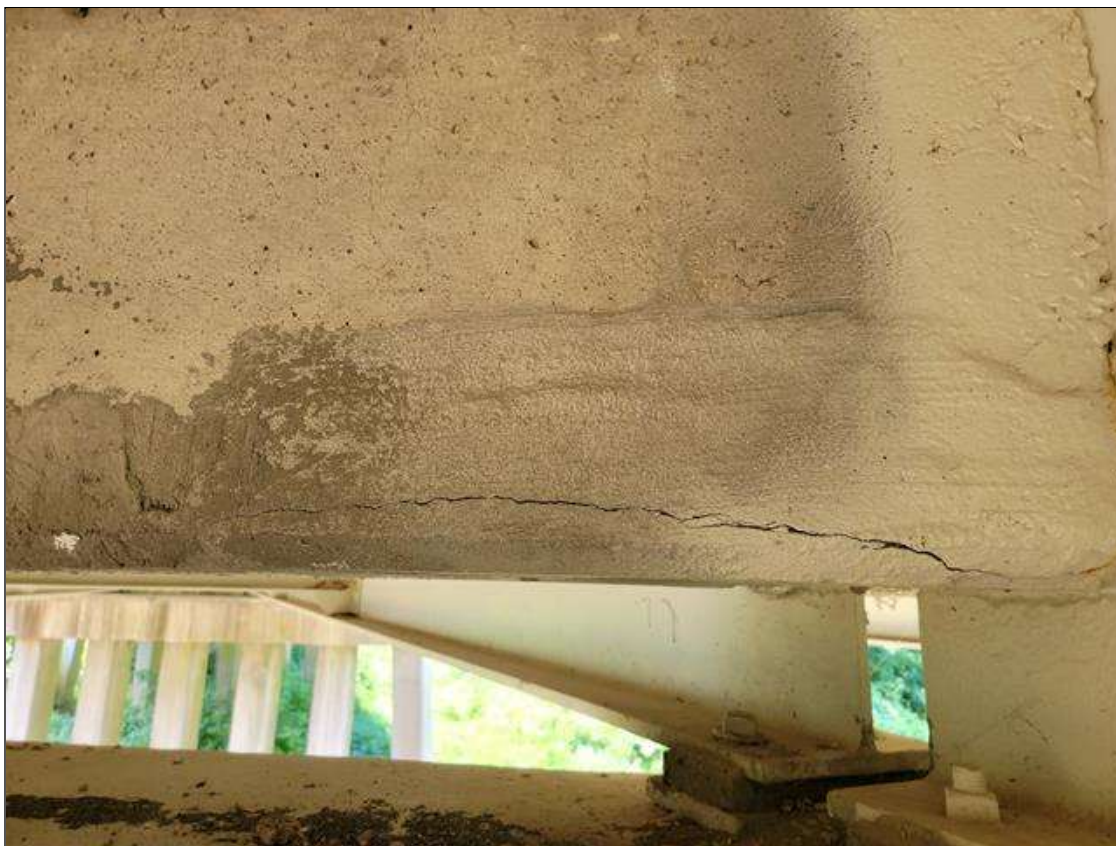
Bent 4 Cap 1: 30 IN LONG X 1/16 IN WIDE HORIZONTAL CRACK, CENTER OF WEST END.
