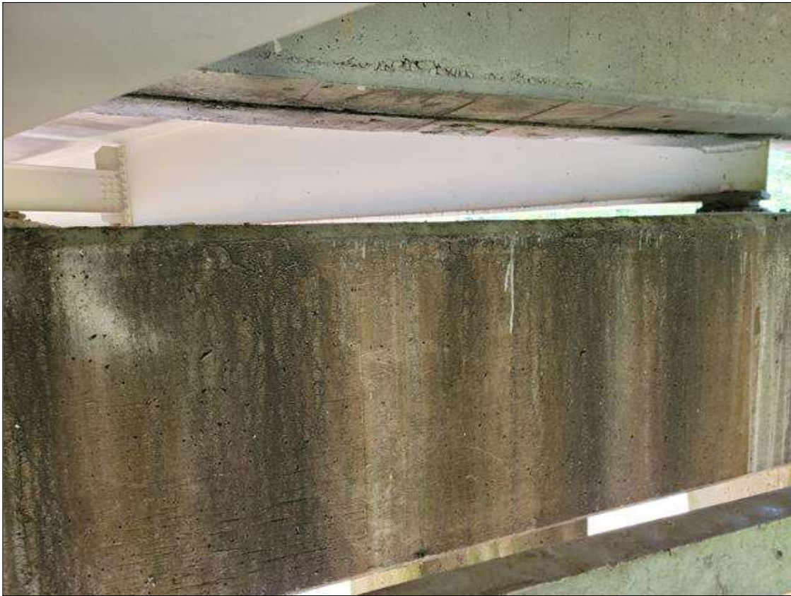
Bent 6 Cap 1: MODERATE LEAKAGE STAINS IN BOTH FACES OF CAP UNDER BEAMS 1 AND 2.
