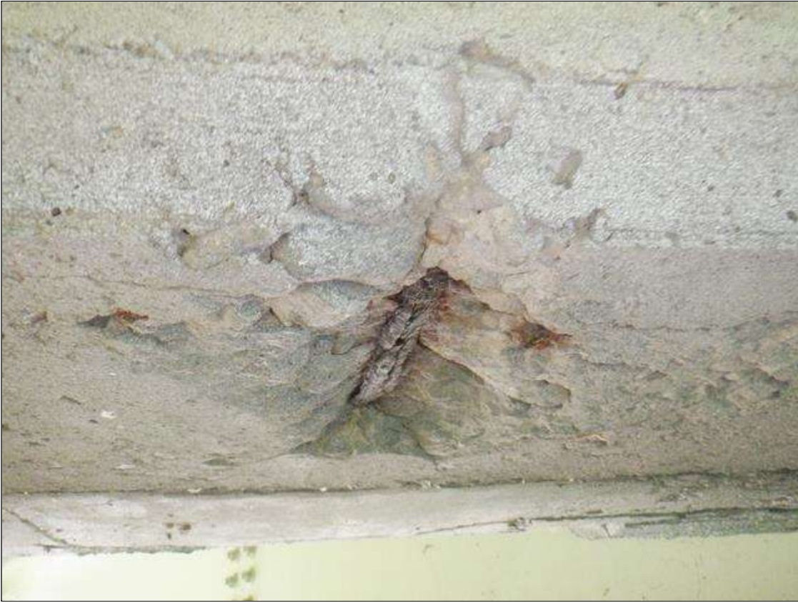
Span 2 Deck: (3) 6 IN DIAMETER X 1/2 IN DEEP SPALLS WITH EXPOSED REINFORCING, UNDERSIDE OF BAY 1 END DIAPHRAGM, AT BENT 2. 90% SECTION REMAINING IN EXPOSED REINFORCING.
