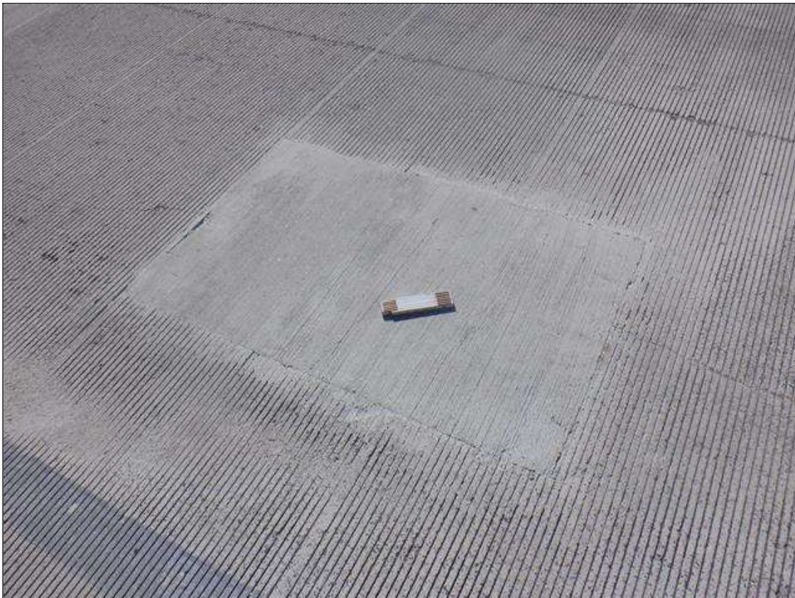
Span 1 Wearing Surface: 4 FT LONG X 3 FT WIDE UNSOUND CONCRETE PATCH WITH 1/16 IN WIDE X 3 FT LONG CRACKS EXTENDING FROM THIS PATCH IN RIGHT LANE AT END BENT 1
