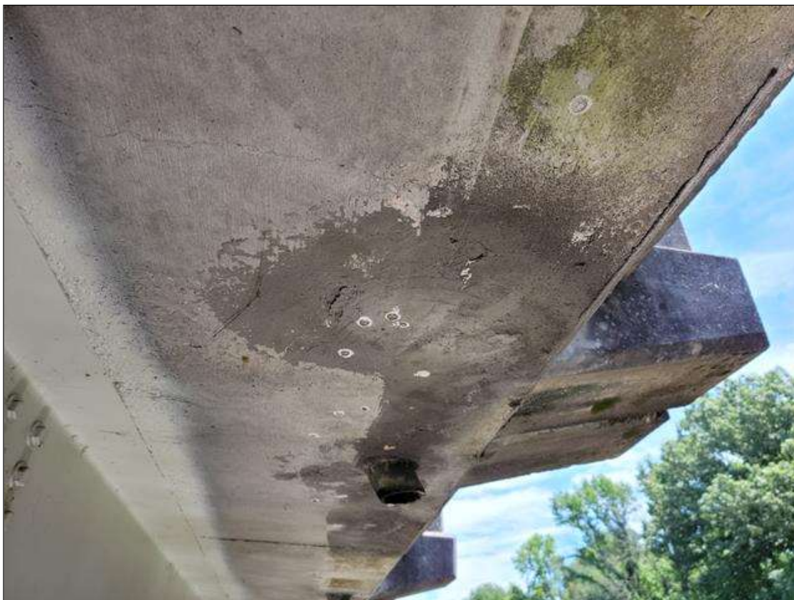
Span 6 Deck: 18 IN DIAMETER SOUND CONCRETE PATCH IN EAST OVERHANG BETWEEN 5TH AND 6TH DECK DRAINS.
