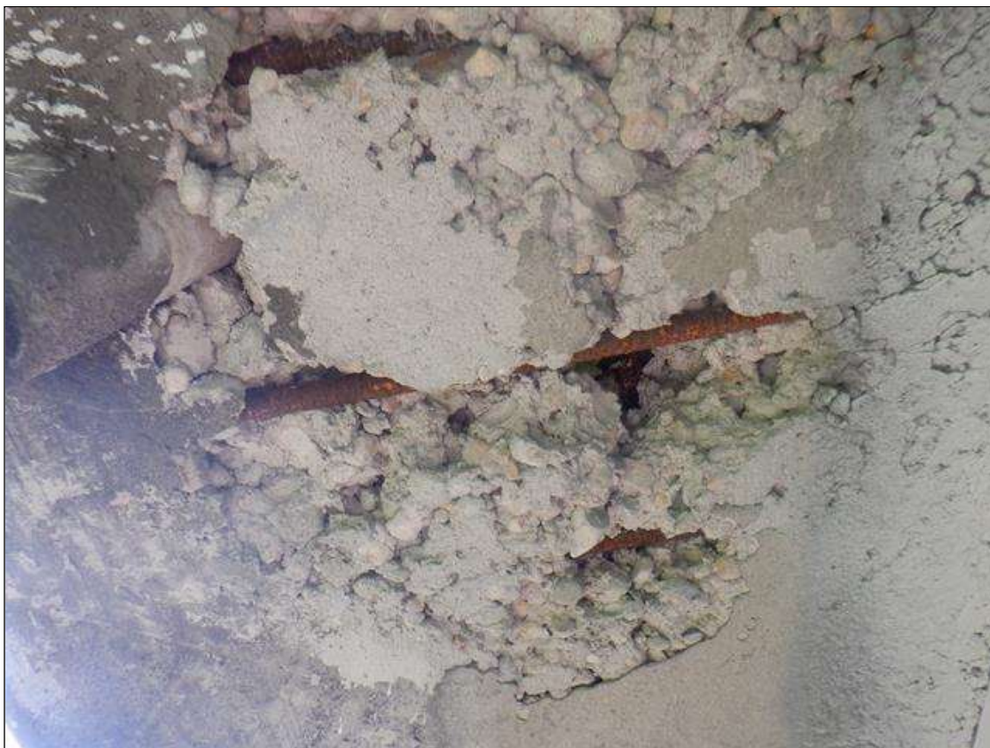
Span 7 Deck: 24 IN LONG X 2 FT WIDE X 2 IN DEEP DELAMINATION/SPALL WITH EXPOSED REINFORCING, UNDERSIDE OF EAST OVERHANG AT 2/3 POINT. 90% REMAINING IN EXPOSED REINFORCEMENT.
