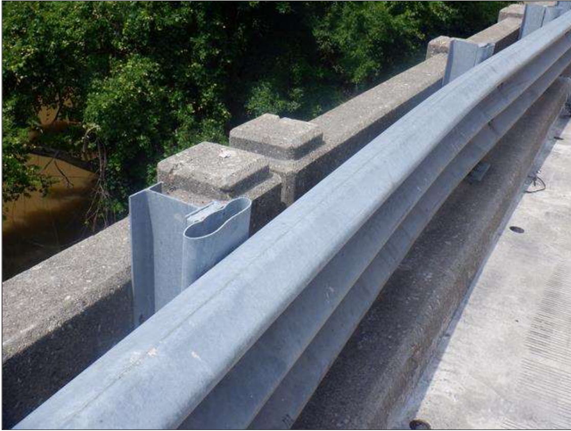
Span 6 Left Bridge Rail: MODERATE TO HEAVY IMPACT DAMAGE WITH UP TO 5 IN DEFLECTION TOWARDS WEST TO THE SUPPLEMENTAL BRIDGE RAIL FOR 20 FT LONG STARTING AT BENT 6. TWO (2) SPACER BLOCKS CONNECTING THE GUARDRAIL TO POSTS ARE PARTIALLY CRUSHED.
