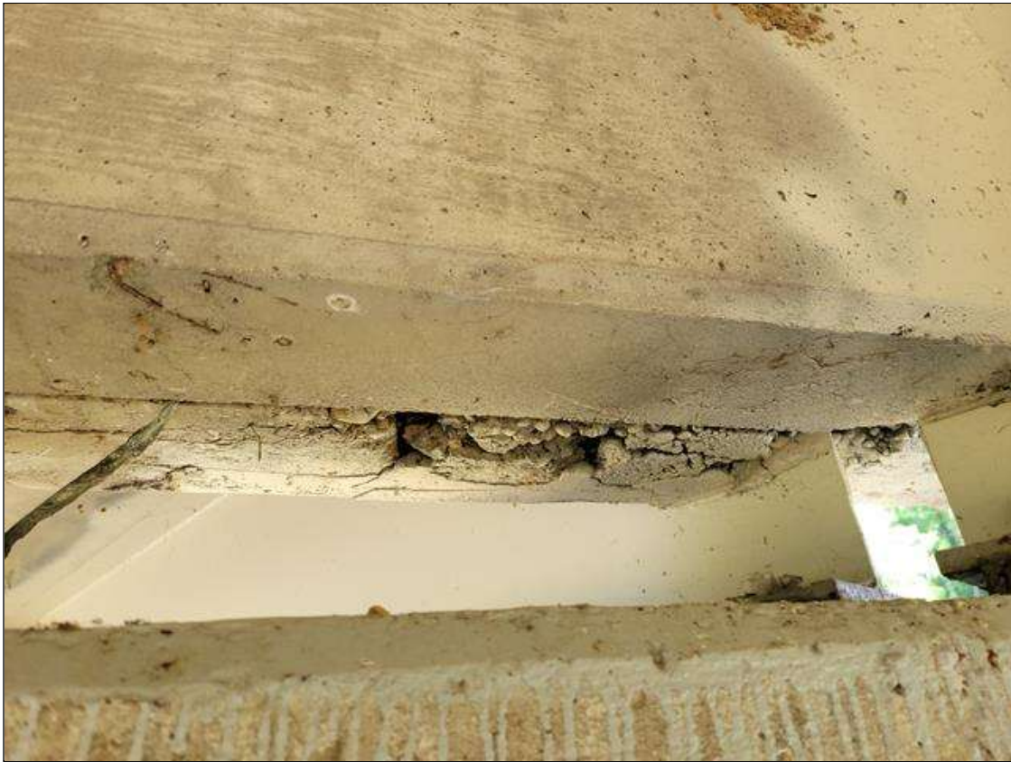
Span 4 Deck: 2 IN WIDE X 7 IN LONG X UP TO 2 IN DEEP SPALLS AND HONEYCOMBING WITH EXPOSED REBAR IN BOTTOM OF DIAPHRAGM IN BAY 1 AT BENT 4. NO MEASUREABLE SECTION LOSS IN EXPOSED REINFORCEMENT.
