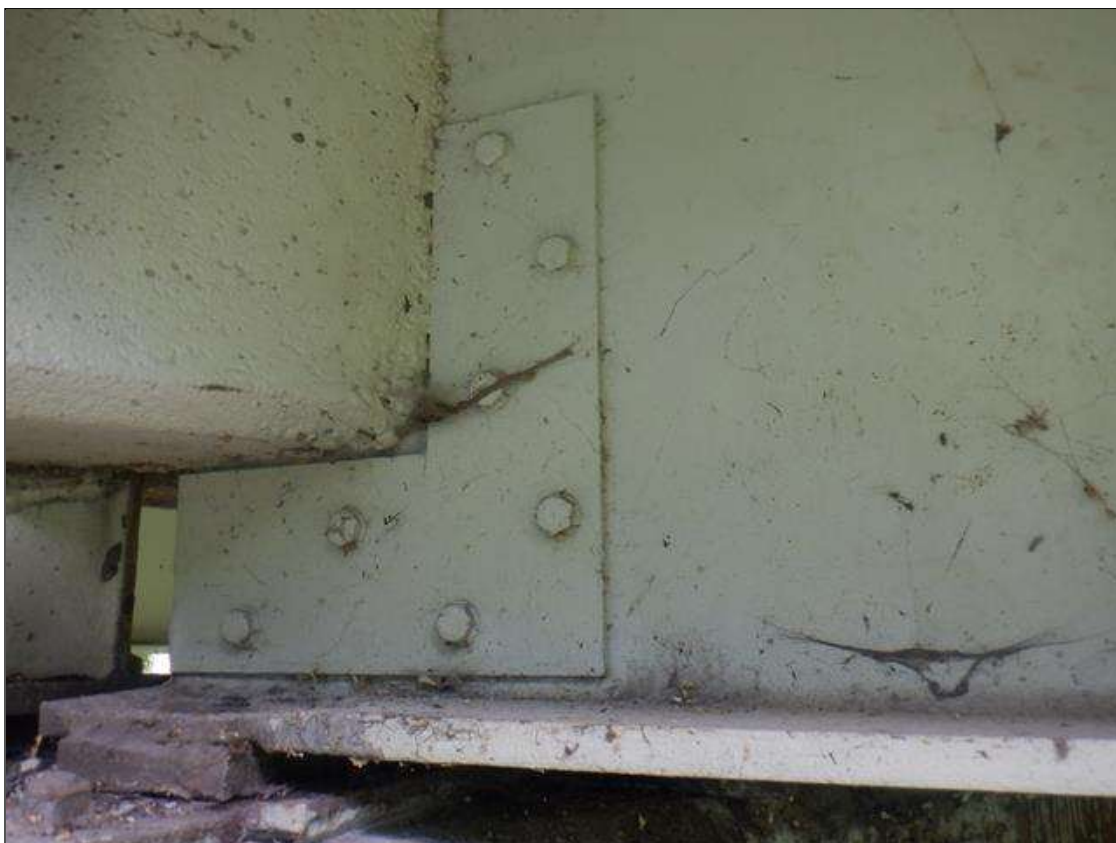
BOLTED PLATE REPAIR TO BOTH SIDES OF WEB FOR BEAM 1 IN SPAN 2 AT BENT 2
