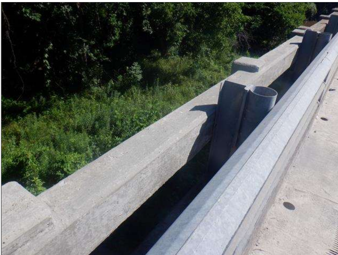
Span 1 Left Bridge Rail: 15 FT LONG AREA OF SOUND CONCRETE PATCHING TO CONCRETE RAIL, BEGINNING AT 15 FT FROM END BENT 1. PREVIOUS REPAIR.
