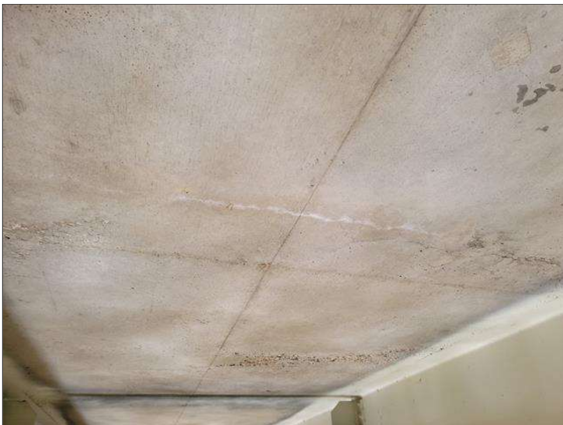
Span 6 Deck: UP TO 0.03 IN WIDE CRACKS IN DECK UNDERSIDE, SCATTERED IN ALL BAYS
