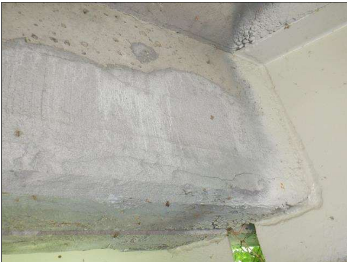
Span 1 Deck: 5 FT WIDE X 1 FT HIGH SOUND CONCRETE PATCH IN BAY 3 END DIAPHRAGM, AT BENT 1. PATCH EXHIBITS A HAIRLINE X 1 FT LONG CRACK IN BOTTOM RIGHT CORNER.
