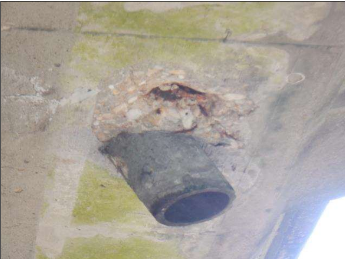
Span 1 Deck: UP TO 6 IN DIAMETER X UP TO 1 IN DEEP SPALL WITH EXPOSED REINFORCEMENT AT THIRD DRAIN PIPE IN LEFT OVERHANG. UP TO 90% SECTION REMAINING IN EXPOSED REINFORCEMENT.
