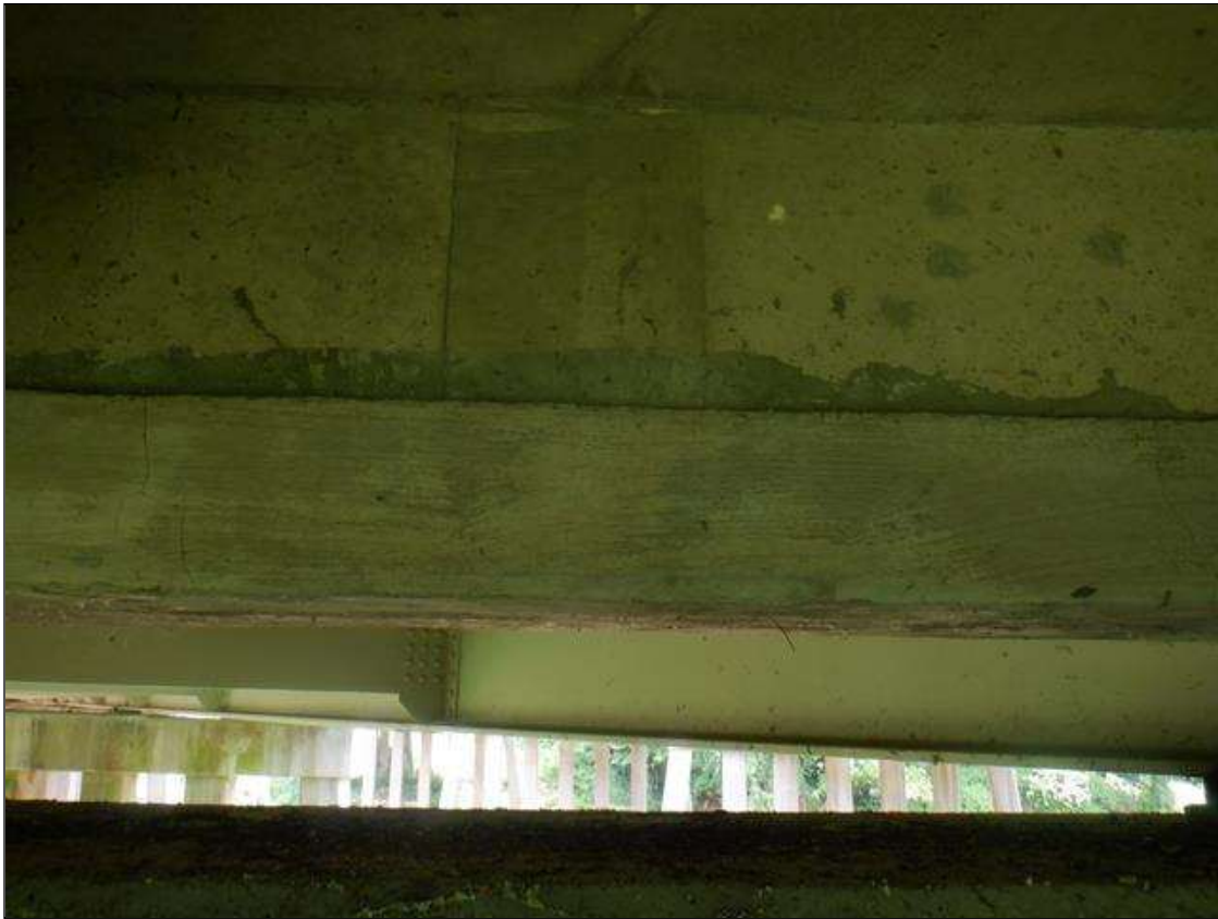
Span 2 Deck: 9 FT LONG X 1 FT HIGH CONCRETE PATCH, BAY 2 END DIAPHRAGM, AT BENT 2. PATCH EXHIBITS UP TO 1/8 IN WIDE X 5 FT LONG CRACK IN THE BOTTOM FACE WITH A 5 FT LONG X 5 IN WIDE UNSOUND CONCRETE AND UP TO 0.02 IN WIDE VERTICAL CRACKS IN FRONT FACE, SCATTERED.
