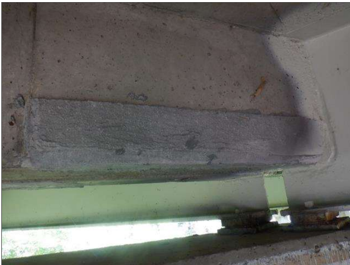
Span 1 Deck: 4 FT LONG X 8 IN HIGH SOUND CONCRETE PATCH IN BAY 2 END DIAPHRAGM, AT BENT 1.
