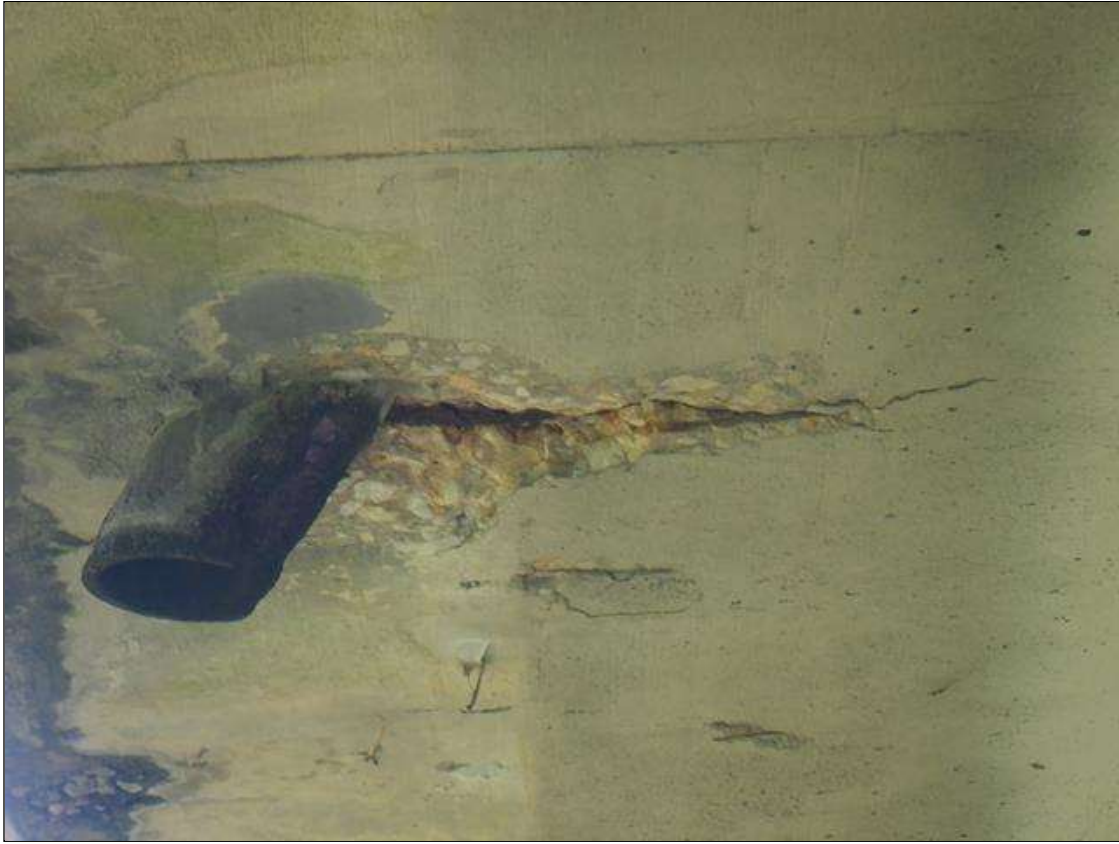
Span 1 Deck: UP TO 1 FT WIDE X 9 IN LONG X UP TO 1 IN DEEP SPALL WITH EXPOSED REINFORCEMENT IN RIGHT OVERHANG, LOCATED AT THIRD DRAIN PIPE. 80% SECTION REMAINING IN EXPOSED REINFORCEMENT.
