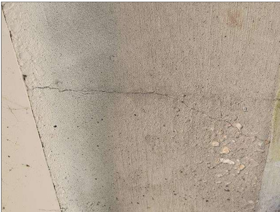
Span 5 Deck: SEVEN (7) UP TO 0.03 IN WIDE X UP TO 3 FT LONG TRANSVERSE CRACKS IN LEFT OVERHANG. TWELVE (12) SIMILAR CRACKS IN RIGHT OVERHANG.
