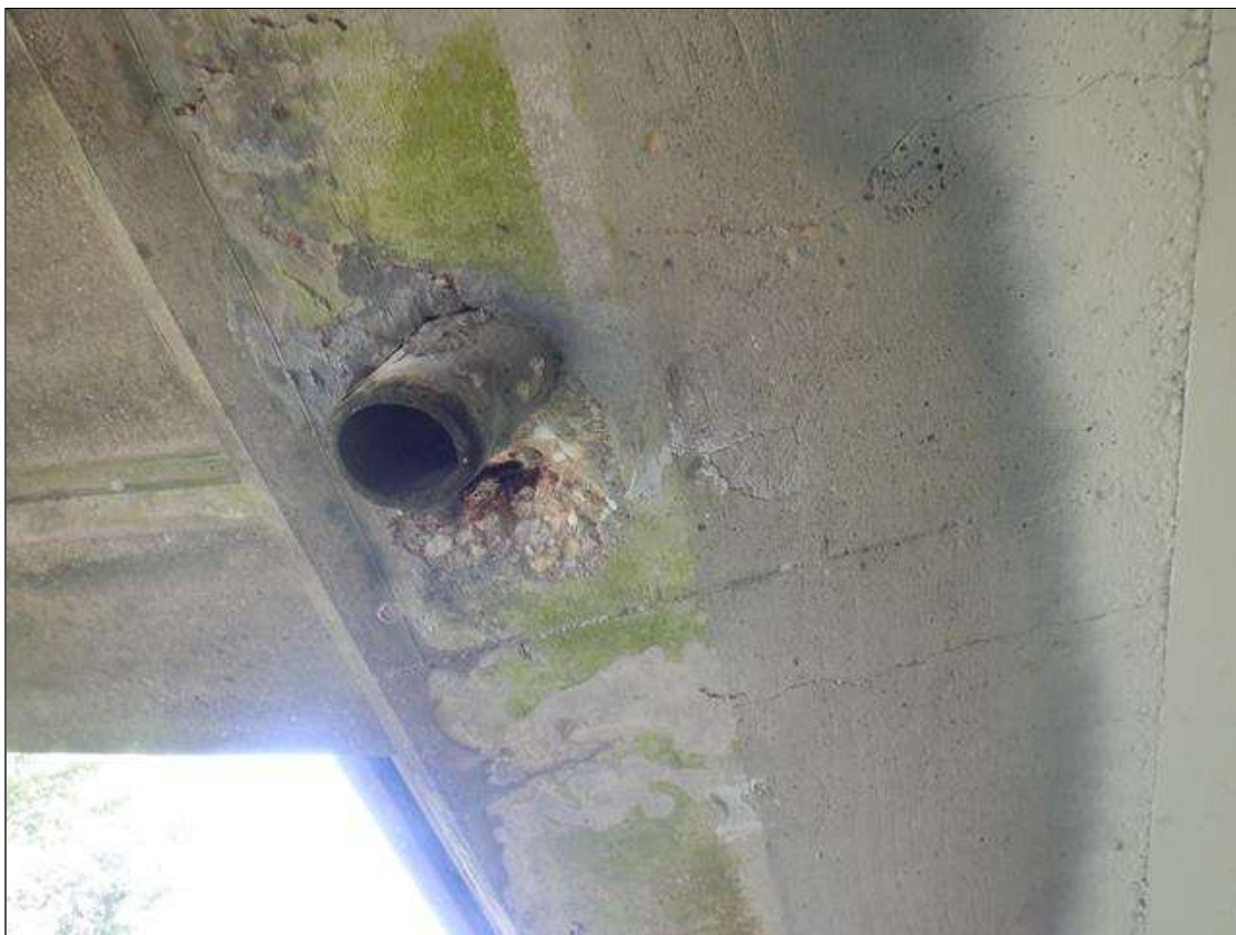
Span 1 Deck: 12 IN DIAMETER X 1.5 IN DEEP SPALL WITH EXPOSED REBAR AT DRAIN 4 IN LEFT OVERHANG. NO MEASURABLE SECTION LOSS IN EXPOSED REBAR.
