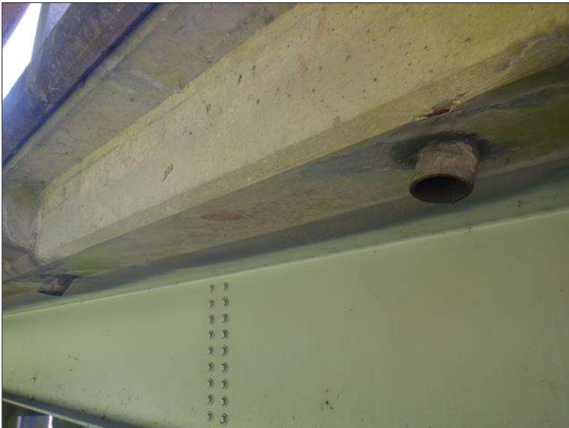
TYPICAL DRAINAGE PIPES UNDER LEFT OVERHANG, SIMILAR UNDER RIGHT OVERHANG
