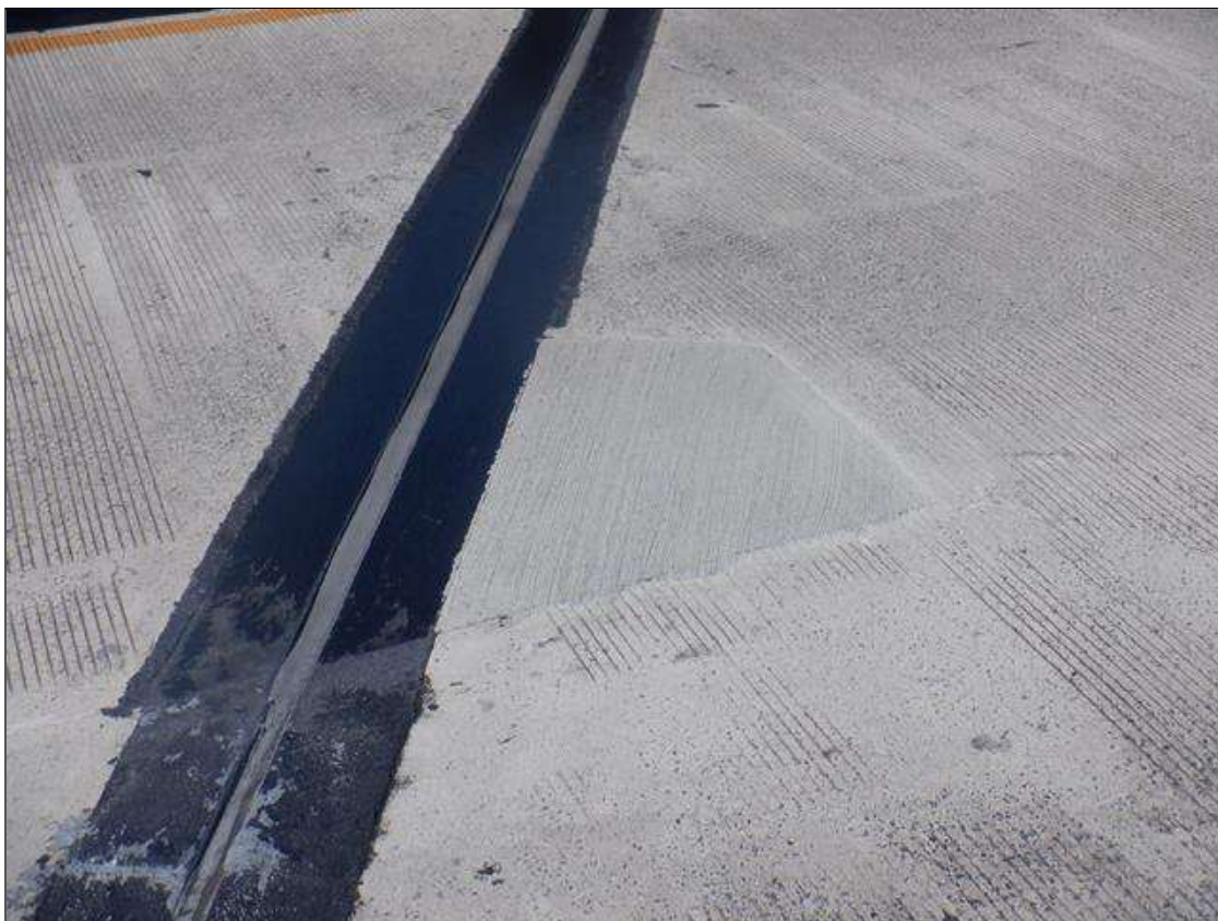
Span 4 Deck: 3 FT LONG X 2 FT WIDE SOUND CONCRETE PATCH IN LEFT TRAVEL LANE AT BENT 4
