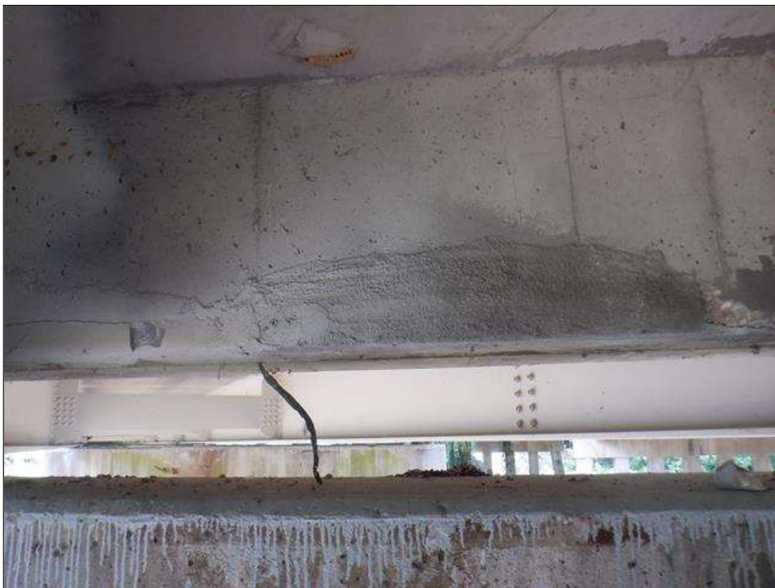
Span 4 Deck: 5 FT LONG X 11 IN HIGH UNSOUND CONCRETE PATCH WITH 1/16 IN WIDE CRACKS AND 2 IN DEEP SPALLS IN BAY 1 AND EXTERIOR END DIAPHRAGM, NEXT TO BEAM 1, AT BENT 4.
