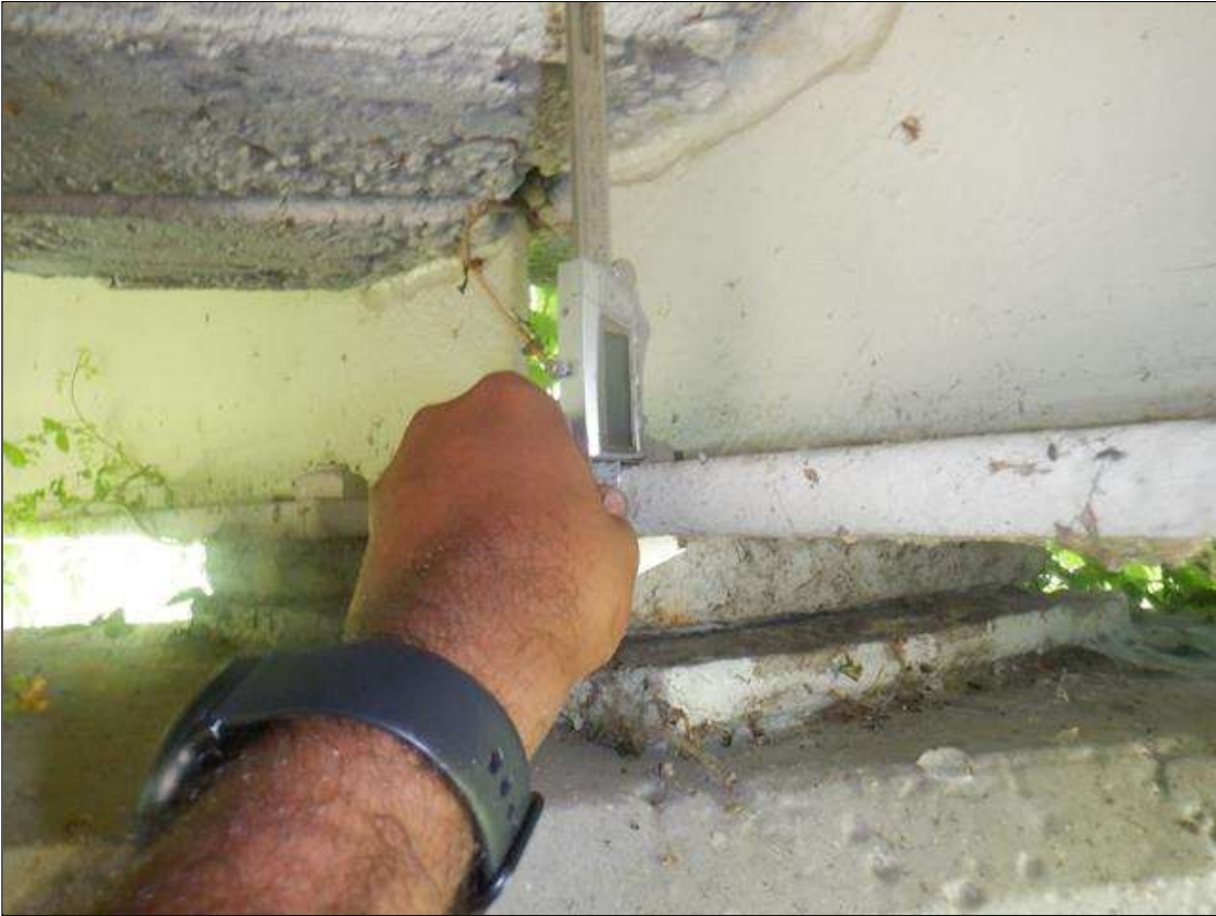
Span 1 Beam 4: 5 IN LONG X 5 IN WIDE AREA OF SECTION LOSS BENEATH THE PAINTED SURFACES IN BOTTOM FLANGE OF LEFT FLANGE ABOVE BEARING AT BENT 1. UP TO 0.77 IN SECTION REMAINING.
