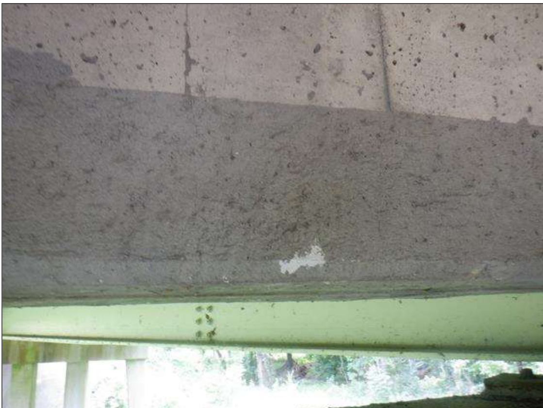
Span 3 Deck: 9 FT LONG X 1 FT HIGH UNSOUND CONCRETE PATCH WITH HAIRLINE CRACKS IN BAY 3 AT BENT 2.
