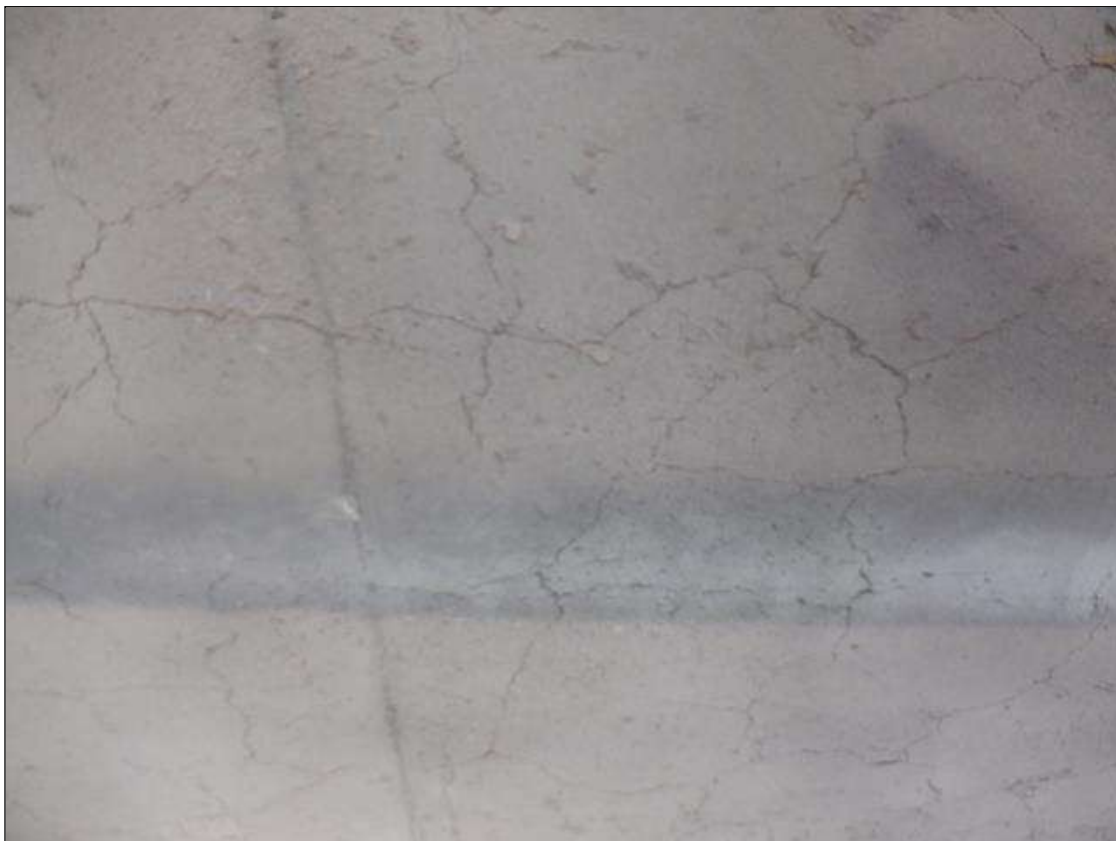
Span 4 Deck: UP TO 0.03 IN WIDE TRANSVERSE AND RANDOM CRACKING IN DECK UNDERSIDE IN ALL BAYS, SCATTERED THROUGHOUT.
