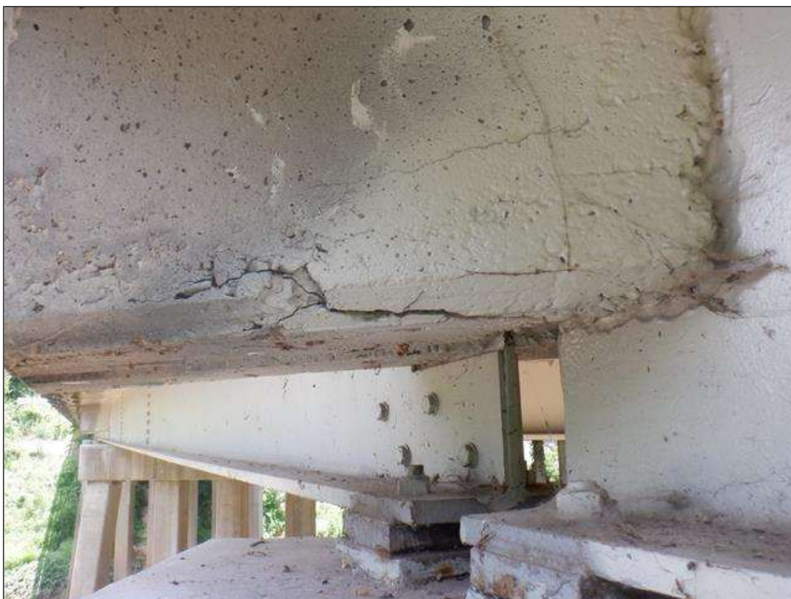
Span 4 Deck: 5 FT LONG X 11 IN HIGH UNSOUND CONCRETE PATCH WITH 1/16 IN WIDE CRACKS AND 2 IN DEEP SPALLS IN BAY 1 AND EXTERIOR END DIAPHRAGM, NEXT TO BEAM 1, AT BENT 4.
