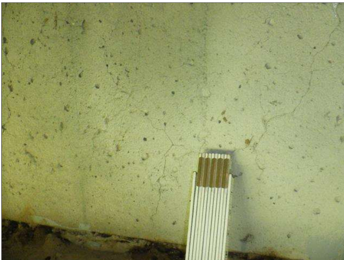
End Bent 1 Abutment: UP TO 0.03 IN WIDE RANDOM CRACKING IN BACKWALL FOR FULL LENGTH.
