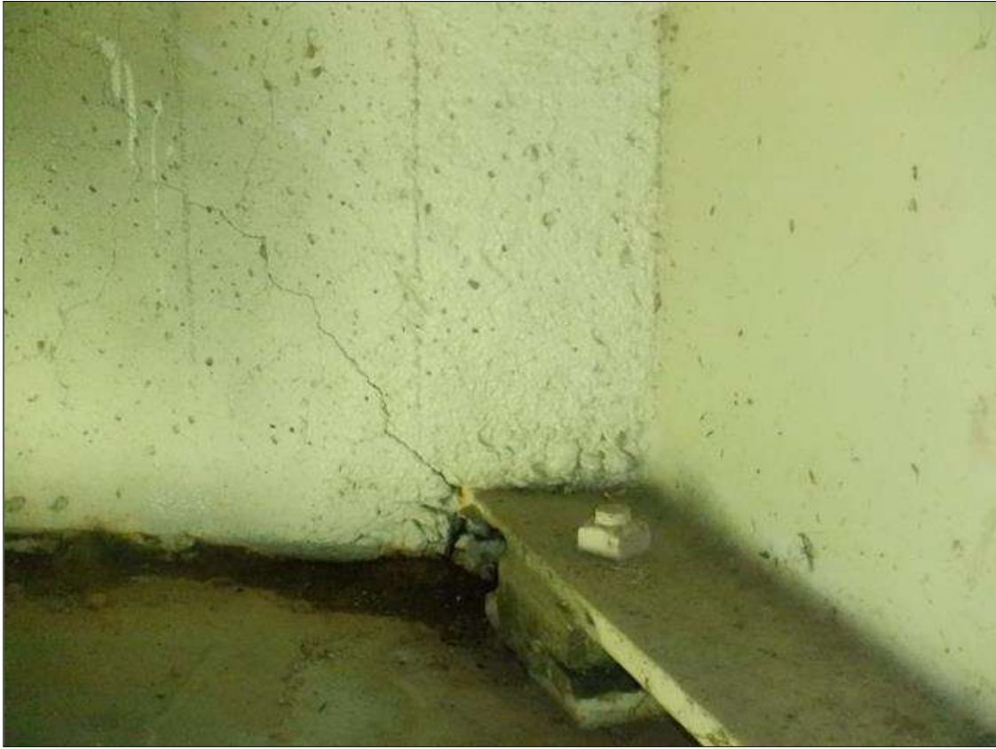
End Bent 1 Abutment: UP TO 1/16 IN WIDE X 2 FT LONG DIAGONAL CRACKS EXTENDING FROM BEARING AT ALL BEAMS
