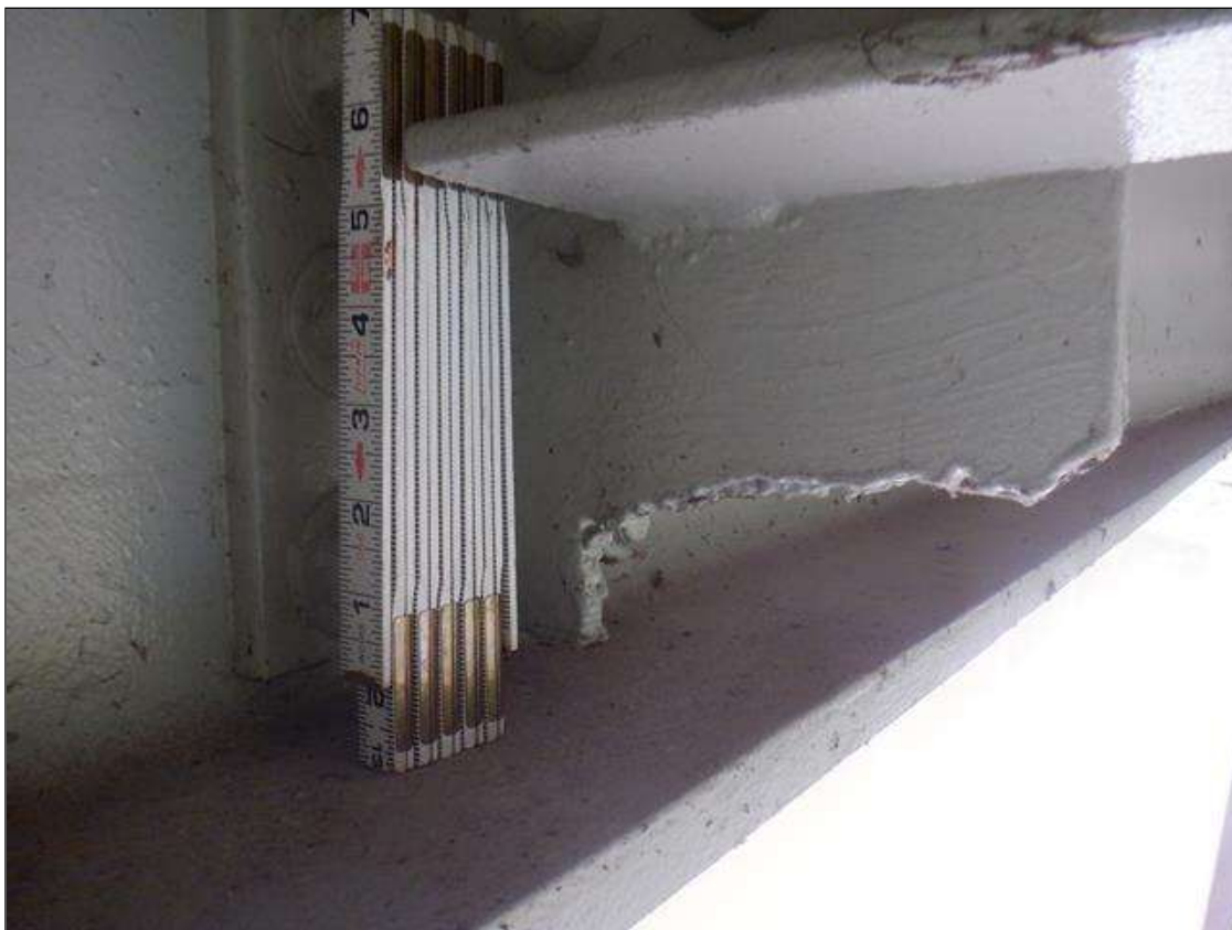
Span 7 Beam 4: UP TO 2 IN HIGH OF SECTION CUT OUT AT BOTTOM OF INTERMEDIATE STIFFENER. PAR IS NOT ISSUED AS IT APPEARS TO BE FROM A BRIDGE REPAIR
