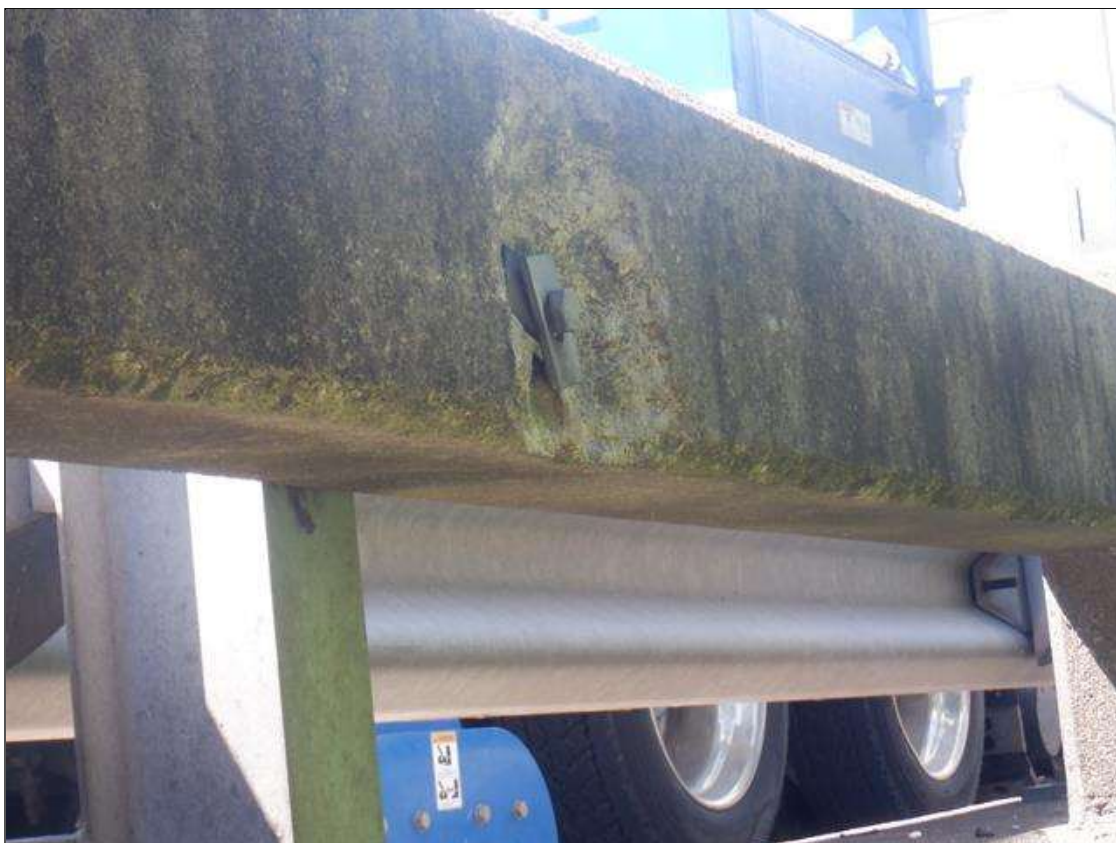
Span 8 Left Bridge Rail: 6 IN DIAMETER X 1.5 IN DEEP SPALL IN ANCHOR BOLT CONNECTION OF SUPPLEMENTAL GUARDRAIL TO BRIDGE RAIL AT SECOND POST FROM END BENT 2
