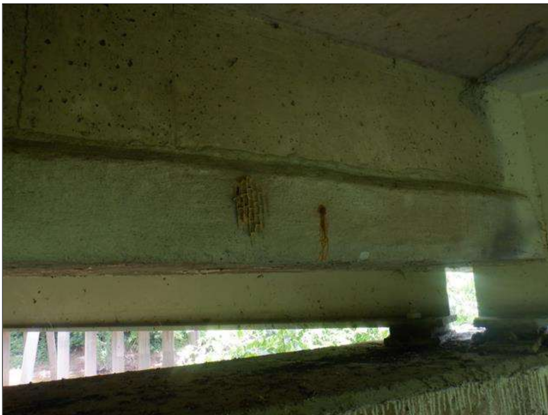
Span 2 Deck: 80 IN LONG X 1 FT HIGH SOUND CONCRETE PATCH IN BAY 3 END DIAPHRAGM, AT BENT 2.
