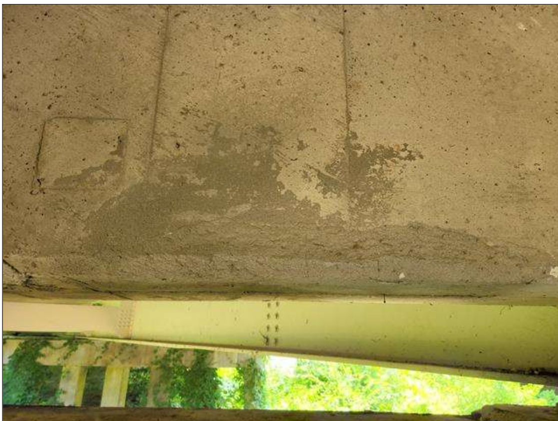
Span 6 Deck: 30 IN LONG X 6 IN HIGH SOUND CONCRETE PATCH IN BAY 1 END DIAPHRAGM, AT BENT 6.
