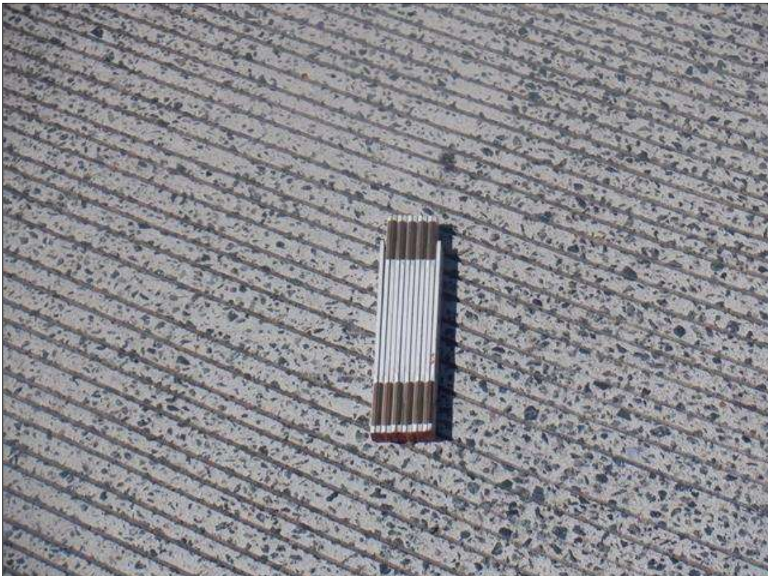
Span 4 Deck: MINOR ABRASION ON WALL MOUNT AND DECK WORN OUT WITH EXPOSED AGGREGATE IN WHEEL PATHS OF BOTH TRAVEL LANES
