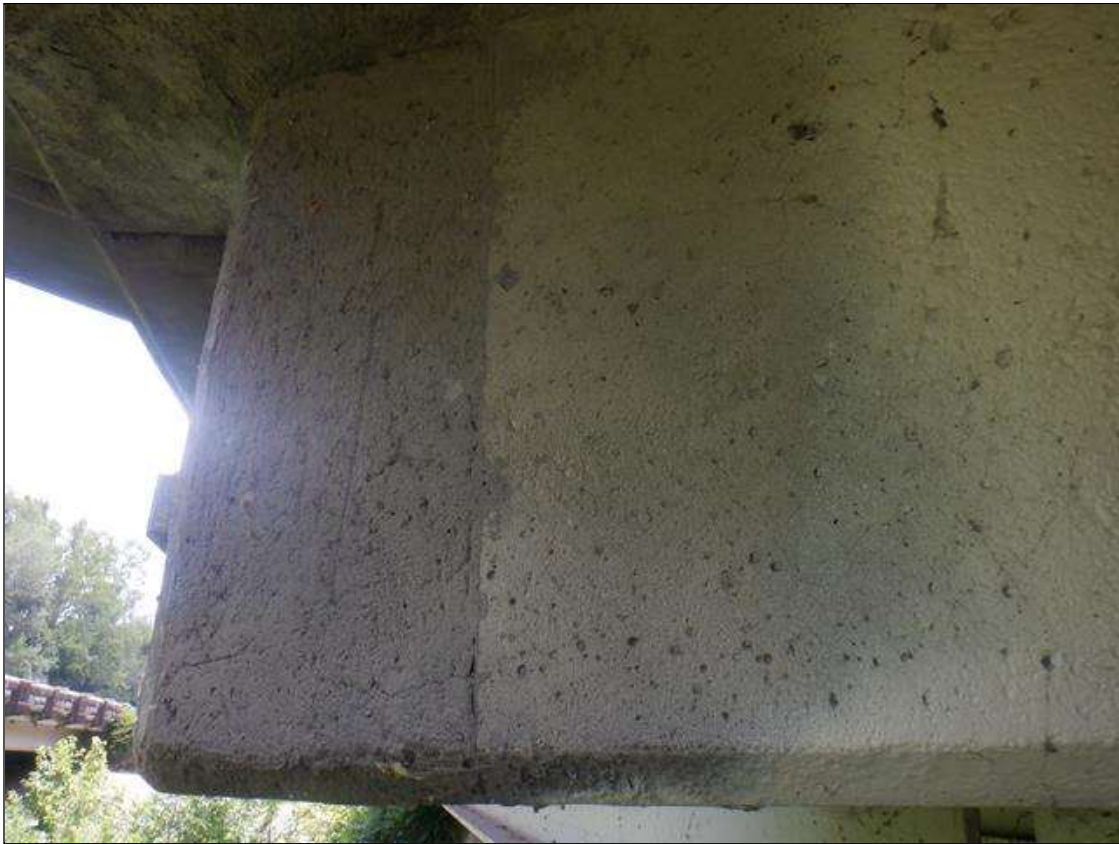
Span 3 Deck: 20 IN HIGH X 1 FT WIDE SOUND CONCRETE PATCH IN EAST OVERHANG AT BENT 2.
