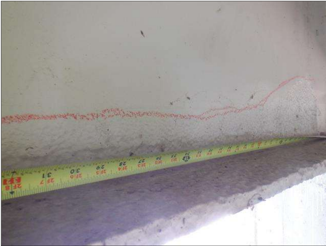
Span 3 Beam 1: 3.3 FT LONG X UP TO 5 IN HIGH AREA OF RIGHT FACE OF THE WEB AT 1.25 FT FROM BEAM END AT BENT 3 EXHIBITS SECTION LOSS BENEATH THE PAINTED SURFACE. UP TO 0.56 IN SECTION REMAINING.
