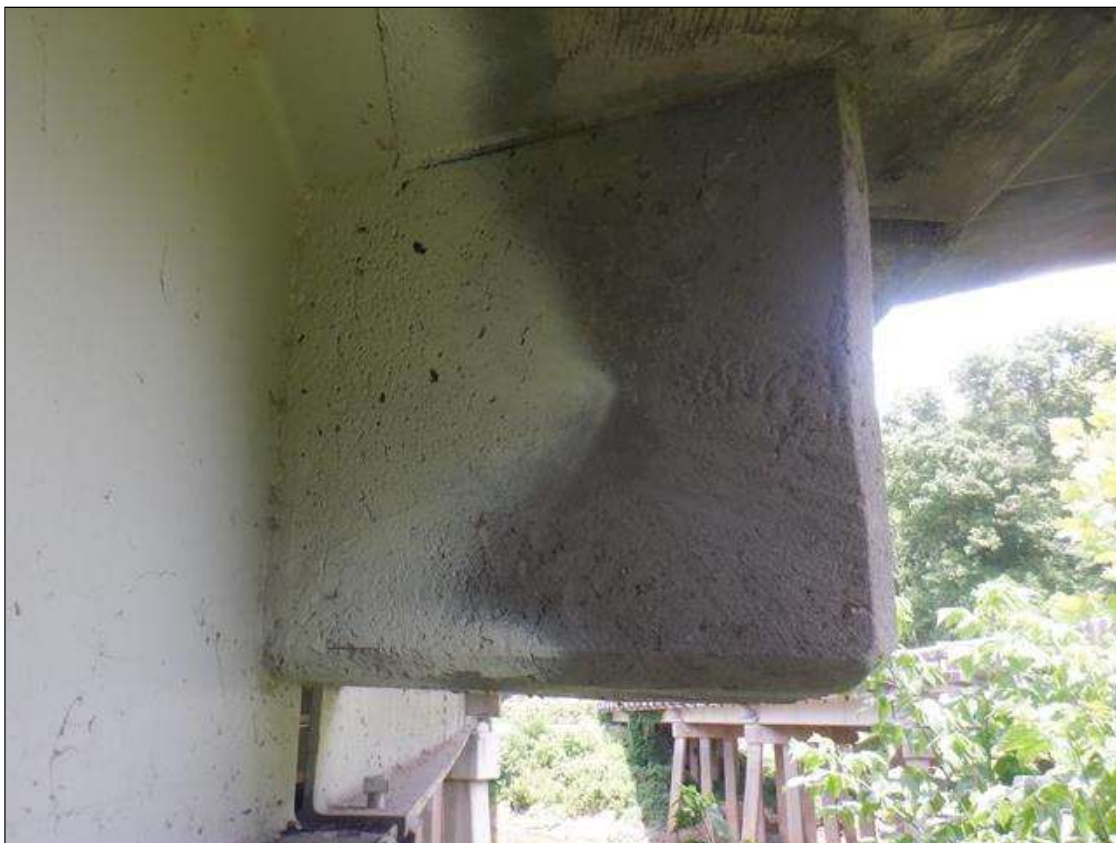
Span 2 Deck: 3 FT WIDE X 1 FT HIGH SOUND CONCRETE PATCH IN OVERHANG IN EAST FACE AT BENT 2 AND A 1 FT WIDE X 2 FT HIGH SOUND CONCRETE PATCH IN DIAPHRAGM OUTSIDE OF BEAM 4 AT BENT 2.
