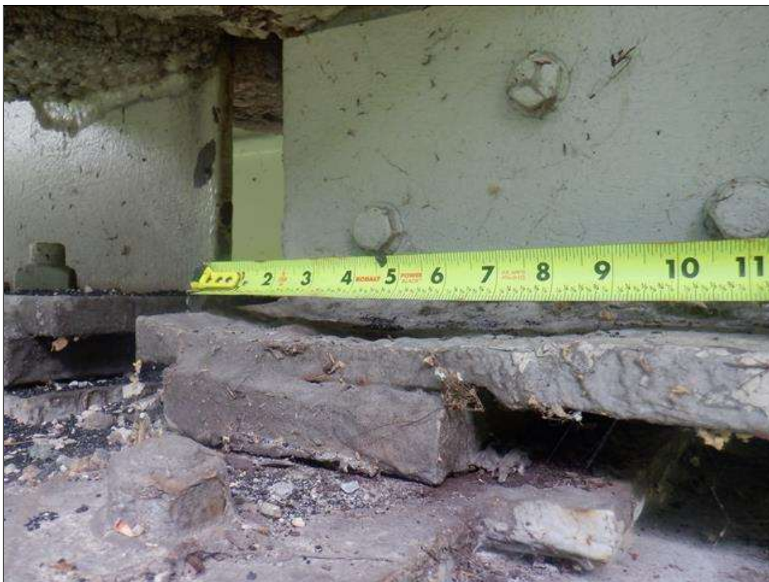
Span 2 Beam 1: 10 IN LONG X 5 IN WIDE AREA OF SECTION LOSS BENEATH THE PAINTED SURFACE ABOVE THE BEARING AT BENT 2. 0.60 IN SECTION REMAINING (PAR).
