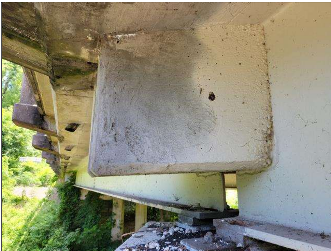
Span 6 Deck: 2 FT HIGH X 1 FT WIDE SOUND CONCRETE PATCH IN END DIAPHRAGM OUTSIDE BEAM 1 AT BEAM 6.
