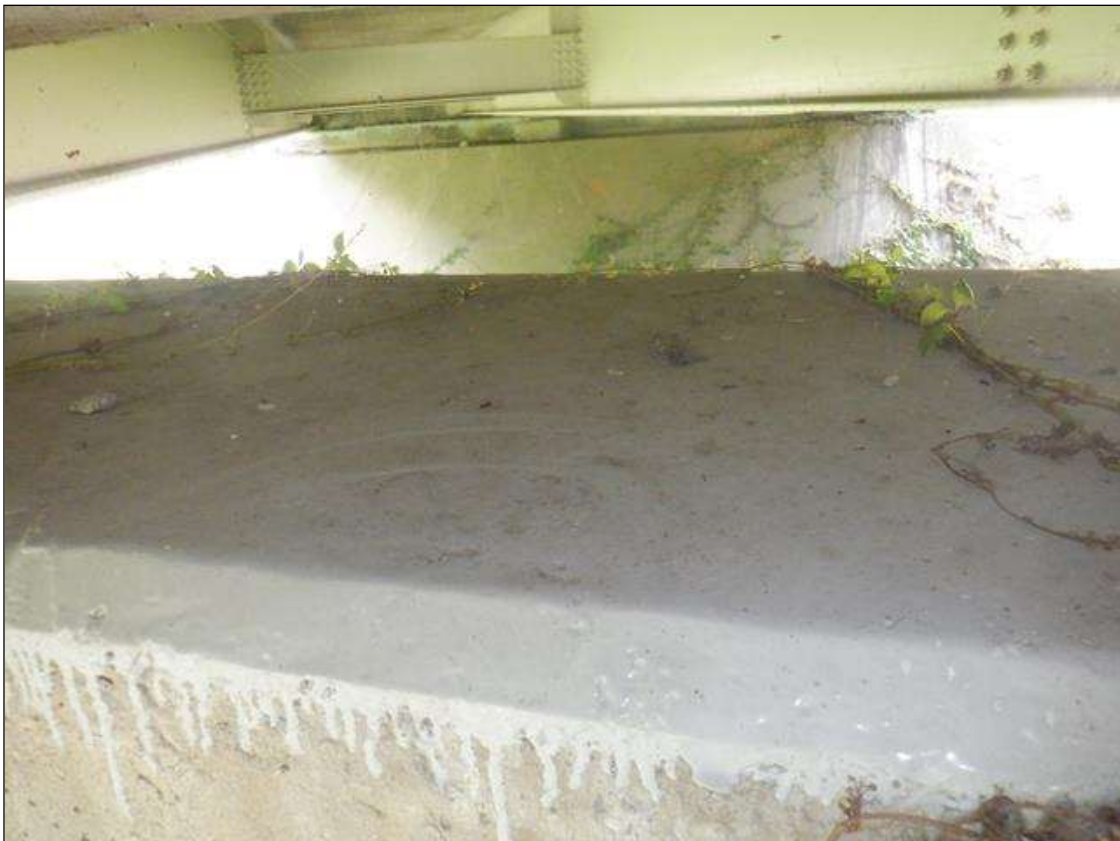
TYPICAL TOP OF BENT CAPS PAINTED OVER
