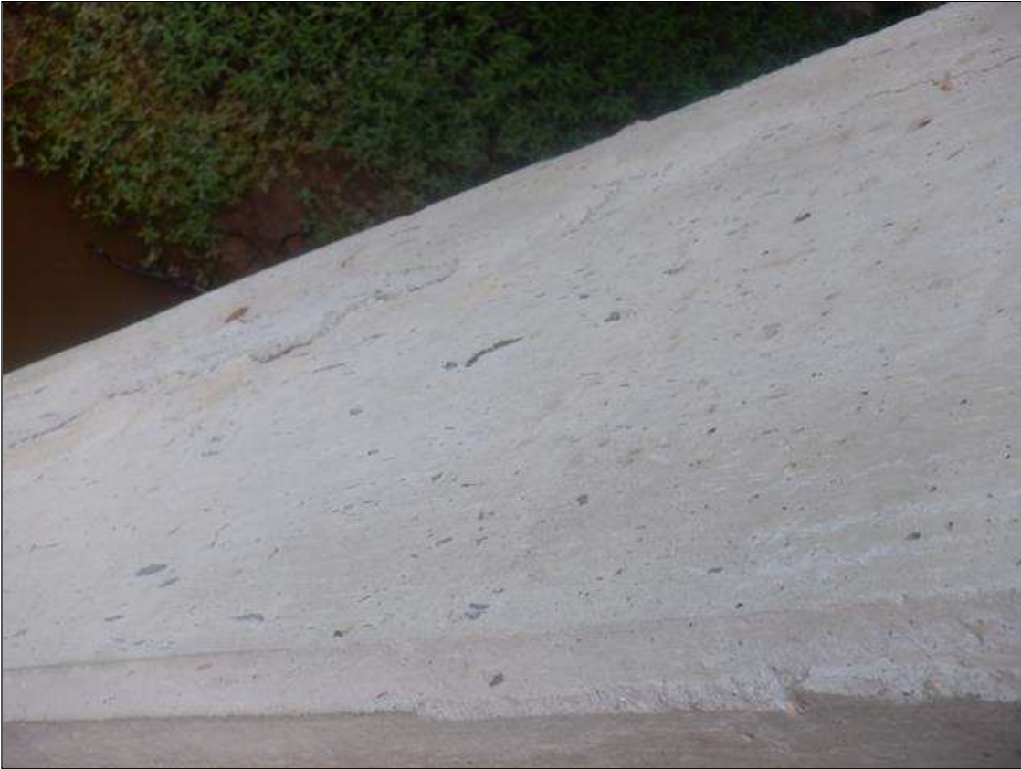
Bent 3 Pile 7: 5 FT HIGH X UP TO 6 IN WIDE CONCRETE PATCH WITH HAIRLINE VERTICAL CRACKS IN EAST FACE, LOCATED AT 4 FT BELOW THE CAP.
