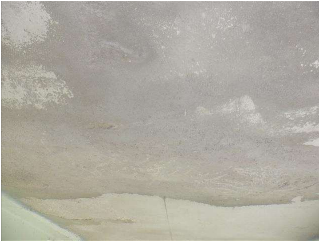
Span 7 Deck: 75 SQ FT OF PATCHED AREA, UNDERSIDE OF DECK, AT RANDOM THROUGHOUT ALL BAYS.
