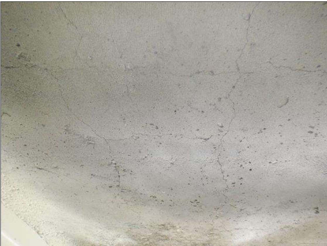
Span 7 Deck: UP TO 0.02 IN WIDE RANDOM CRACKING IN DECK UNDERSIDE IN ALL BAYS, SCATTERED THROUGHOUT.
