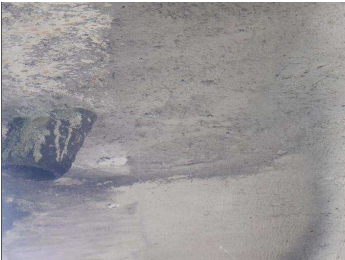
Span 7 Deck: 18 IN DIAMETER SOUND CONCRETE PATCH IN EAST OVERHANG AT THIRD DRAIN PIPE.
