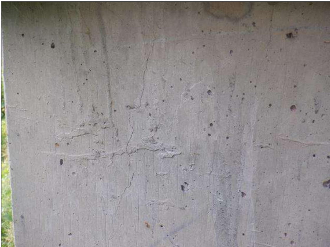
Bent 2 Pile 7: UP TO 0.05 IN WIDE X 22 IN HIGH VERTICAL CRACK IN TOP OF NORTH FACE.
