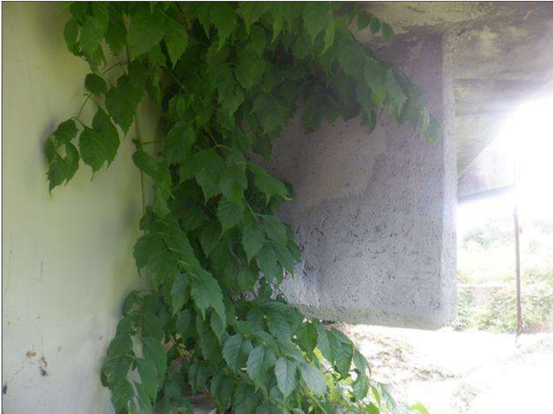
Span 7 Deck: 2 FT HIGH X 1 FT WIDE SOUND CONCRETE PATCH IN DIAPHRAGM OUTSIDE BEAM 4 AT BENT 7.
