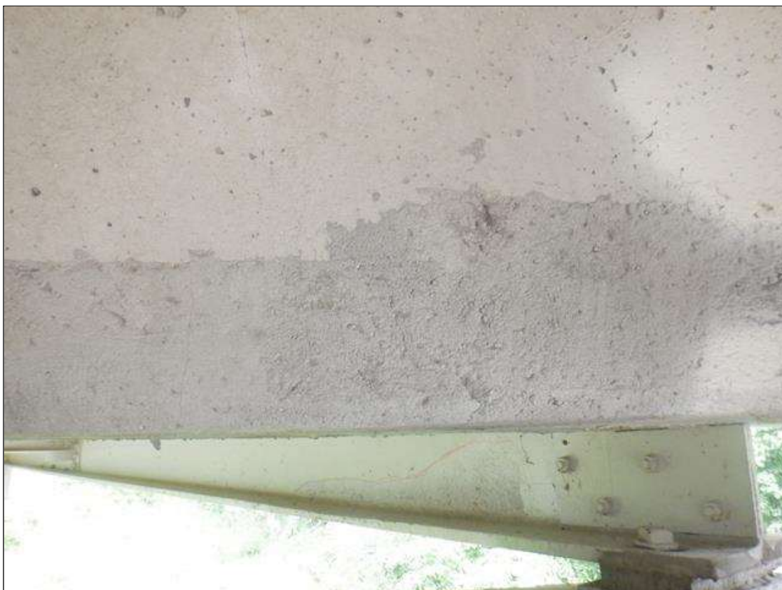
Span 4 Deck: 2.5 FT LONG X 6 IN HIGH SOUND CONCRETE PATCH WITH HAIRLINE VERTICAL CRACKS IN BAY 1 ABOVE BENT 3.
