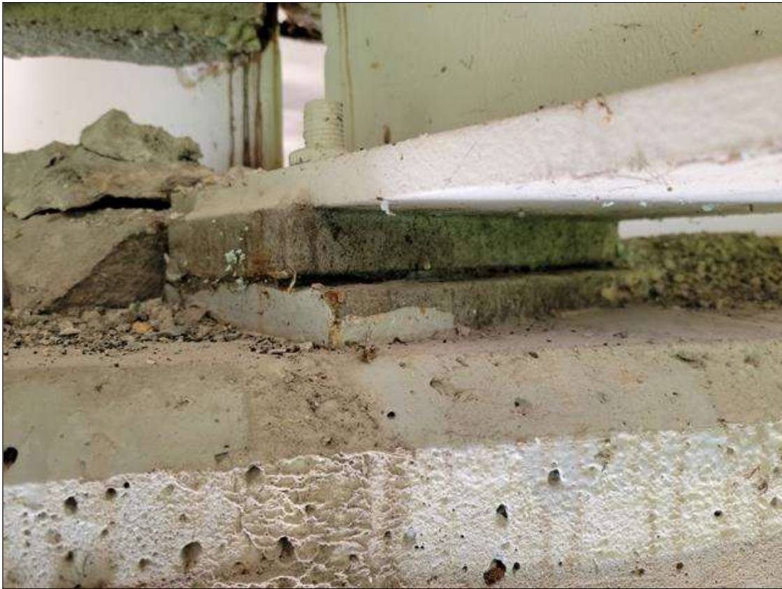
Span 7 Near Bearing: BEARINGS HAVE BEEN PAINTED SINCE PREVIOUS INSPECTION. SECTION LOSS REMAINS BENEATH THE PAINTED SURFACES. UP TO 90% SECTION REMAINING IN BOTH MASONRY AND SOLE PLATES.
