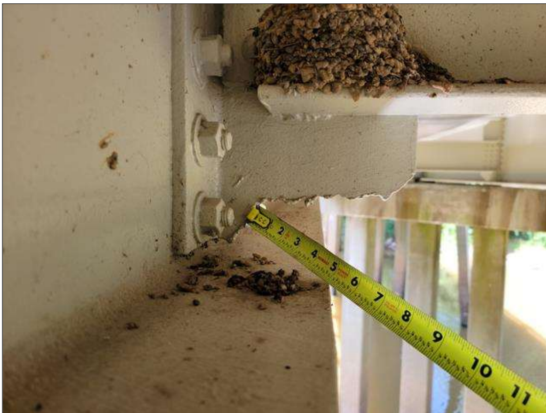
Span 6 Beam 4: UP TO 2 IN HIGH OF SECTION CUT OUT AT BOTTOM OF INTERMEDIATE STIFFENER. PAR IS NOT ISSUED AS IT APPEARS TO BE FROM A BRIDGE REPAIR
