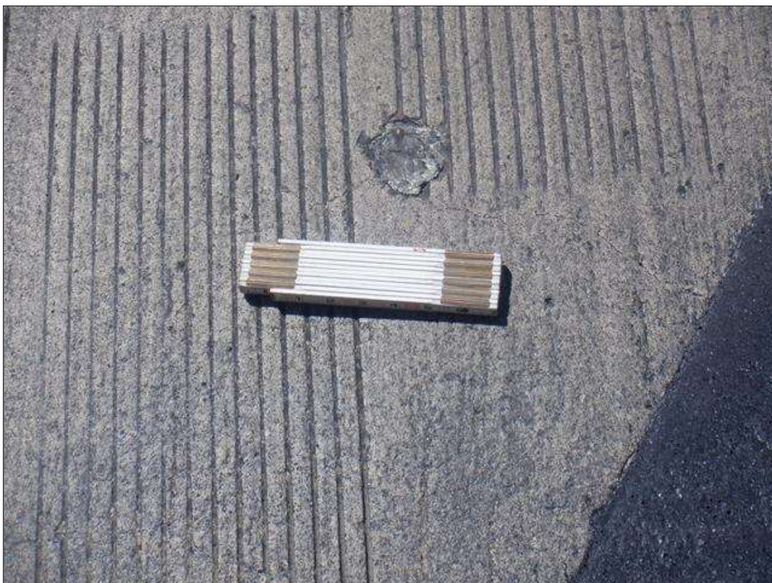
Approach 2 Approach 2: UP TO 0.05 IN WIDE DIAGONAL AND LONGITUDINAL CRACKS IN BOTH TRAVEL LANES
