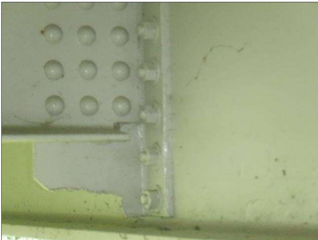
Span 2 Beam 1: UP TO 2 IN HIGH OF SECTION CUT OUT AT BOTTOM OF INTERMEDIATE STIFFENER. PAR IS NOT ISSUED AS IT APPEARS TO BE FROM A BRIDGE REPAIR
