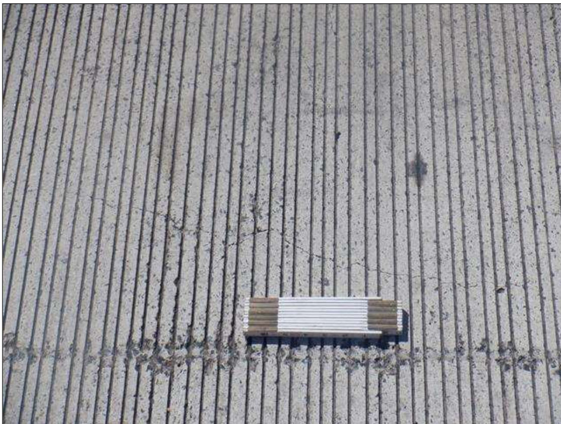
Span 5 Deck: UP TO 0.05 IN WIDE LONGITUDINAL AND TRANSVERSE CRACKS AT MID-SPAN IN BOTH TRAVEL LANES
