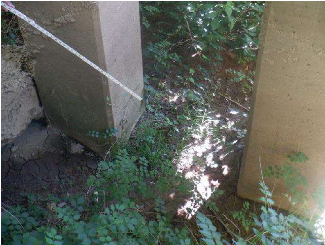
UP TO 2 FT OF EROSION ALONG ALL PILES AT BENT 1
