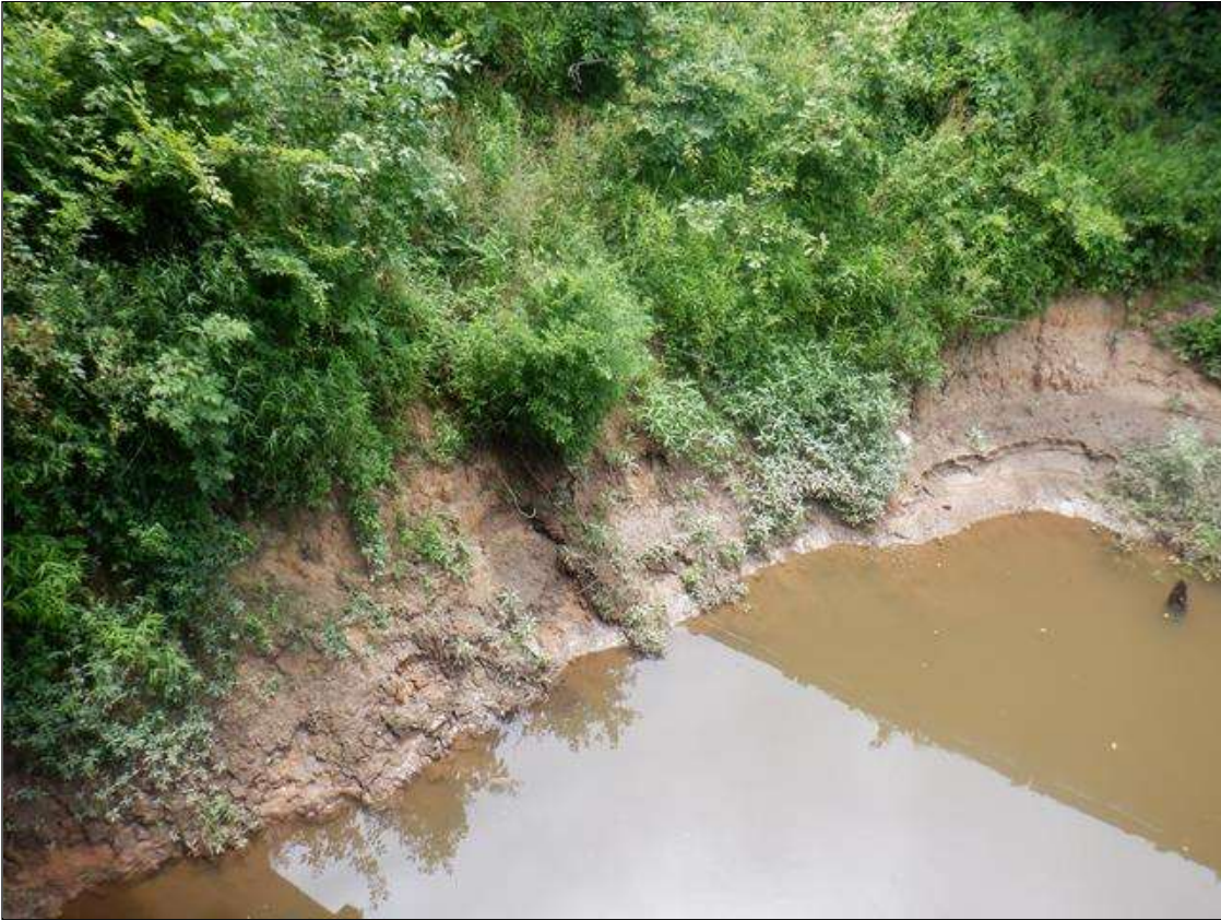
30 FT LONG X 75 FT WIDE X UP TO 10 FT HIGH AREA OF BANK SLOPE EROSION UNDER SPAN 7 AT BENT 7
