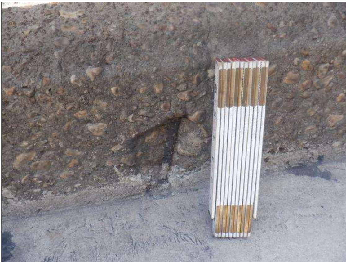
Span 5 Left Bridge Rail: 6 IN DIAMETER X 1 IN DEEP SPALL WITH EXPOSED PAINTED REBAR IN BOTTOM OF CURB AT 3 FT FROM BENT 6 JOINT. 90% SECTION LOSS IN EXPOSED REINFORCEMENT
