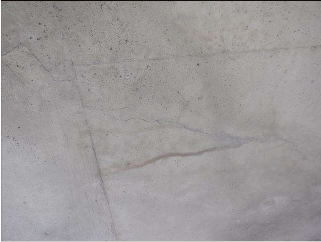
Span 3 Deck: 7 FT LONG X 0.05 IN WIDE DIAGONAL CRACK IN UNDERSIDE OF DECK, BAY 3 AT BENT 2.
