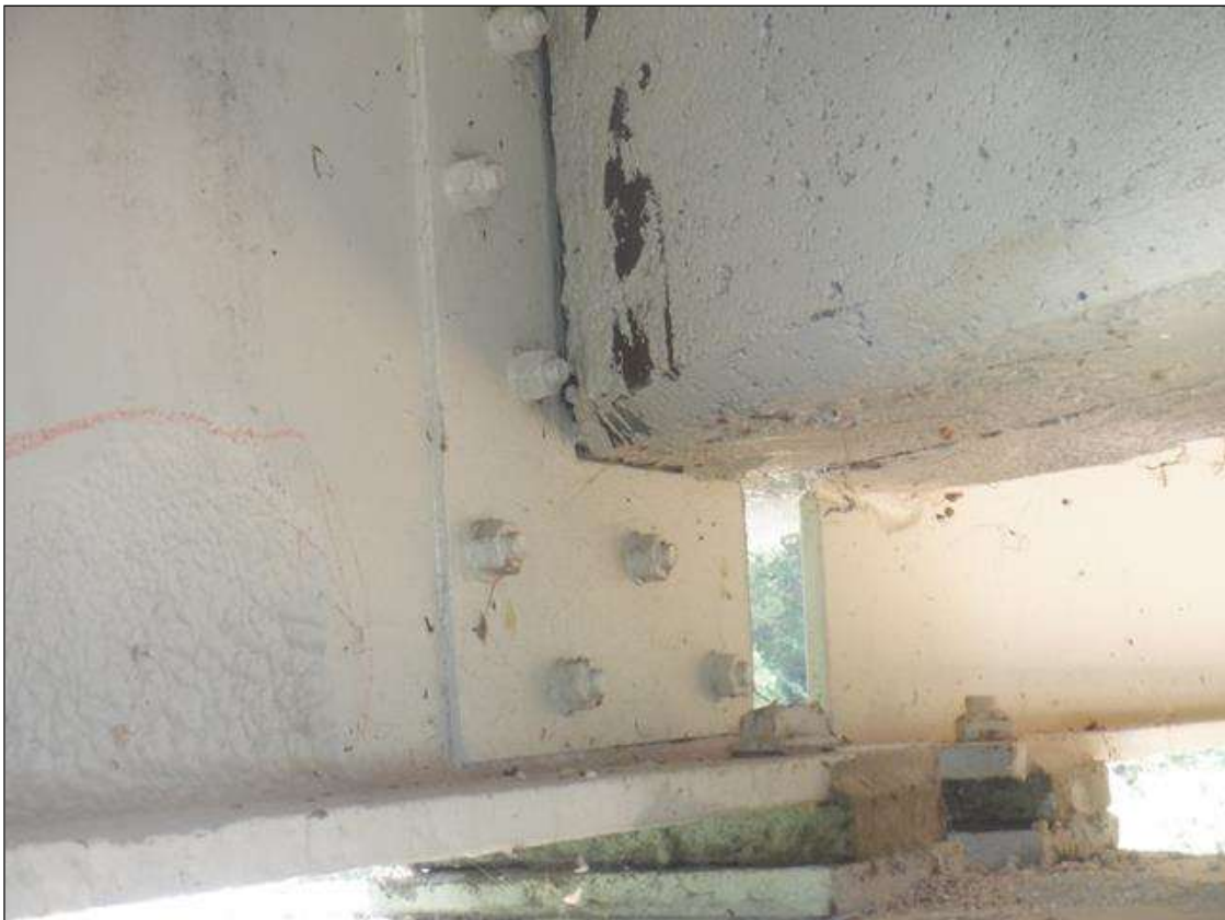
BOLTED PLATE REPAIR TO BOTH SIDES OF WEB FOR BEAM 1 IN SPAN 3 AT BENT 3
