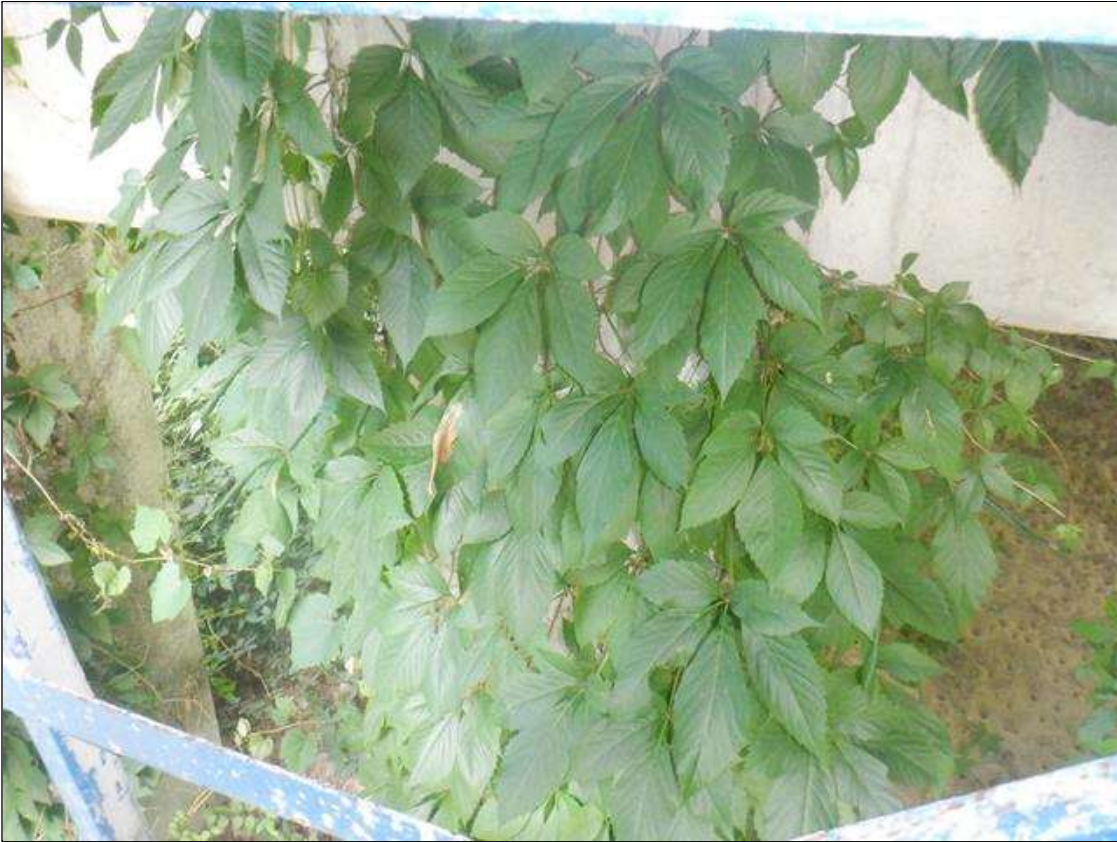
Bent 7 Pile 2: HEAVY VEGETATION GROWTH FOR FULL HEIGHT
