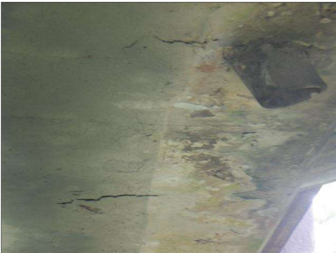
Span 1 Deck: (2) 12 IN DIAMETER DELAMINATIONS, UNDERSIDE OF WEST OVERHANG, AT DRAIN 7.
