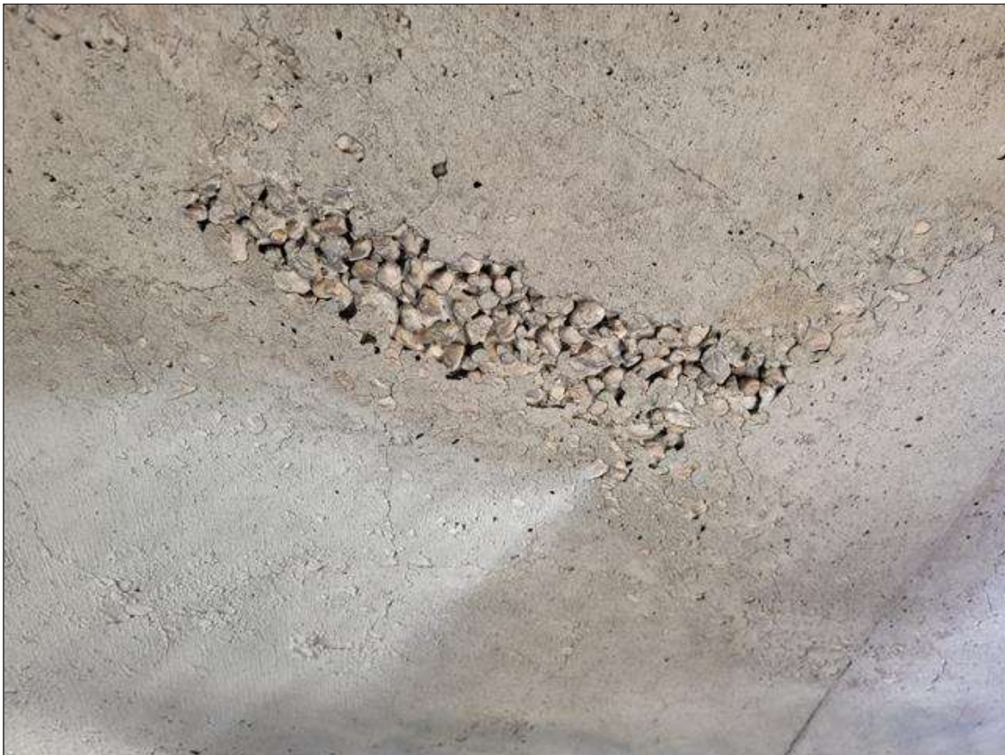
Span 6 Deck: SCATTERED AREAS OF HONEYCOMBING IN DECK UNDERSIDE IN ALL BAYS
