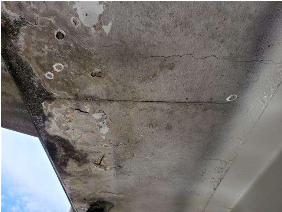
Span 6 Deck: THREE (3) AREAS OF DELAMINATED CONCRETE UP TO 6 IN DIAMETER IN EAST OVERHANG AT BENT 6.
