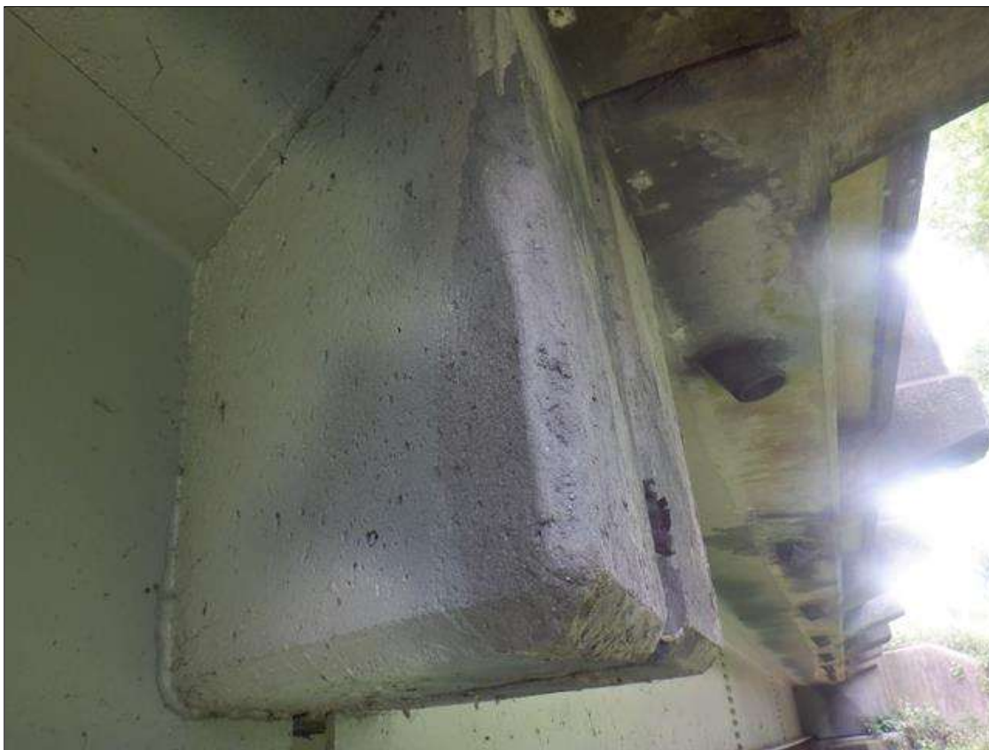
Span 2 Deck: 1 FT DIAMETER SOUND CONCRETE PATCH IN DIAPHRAGM OUTSIDE OF BEAM 1 AT BENT 1.
