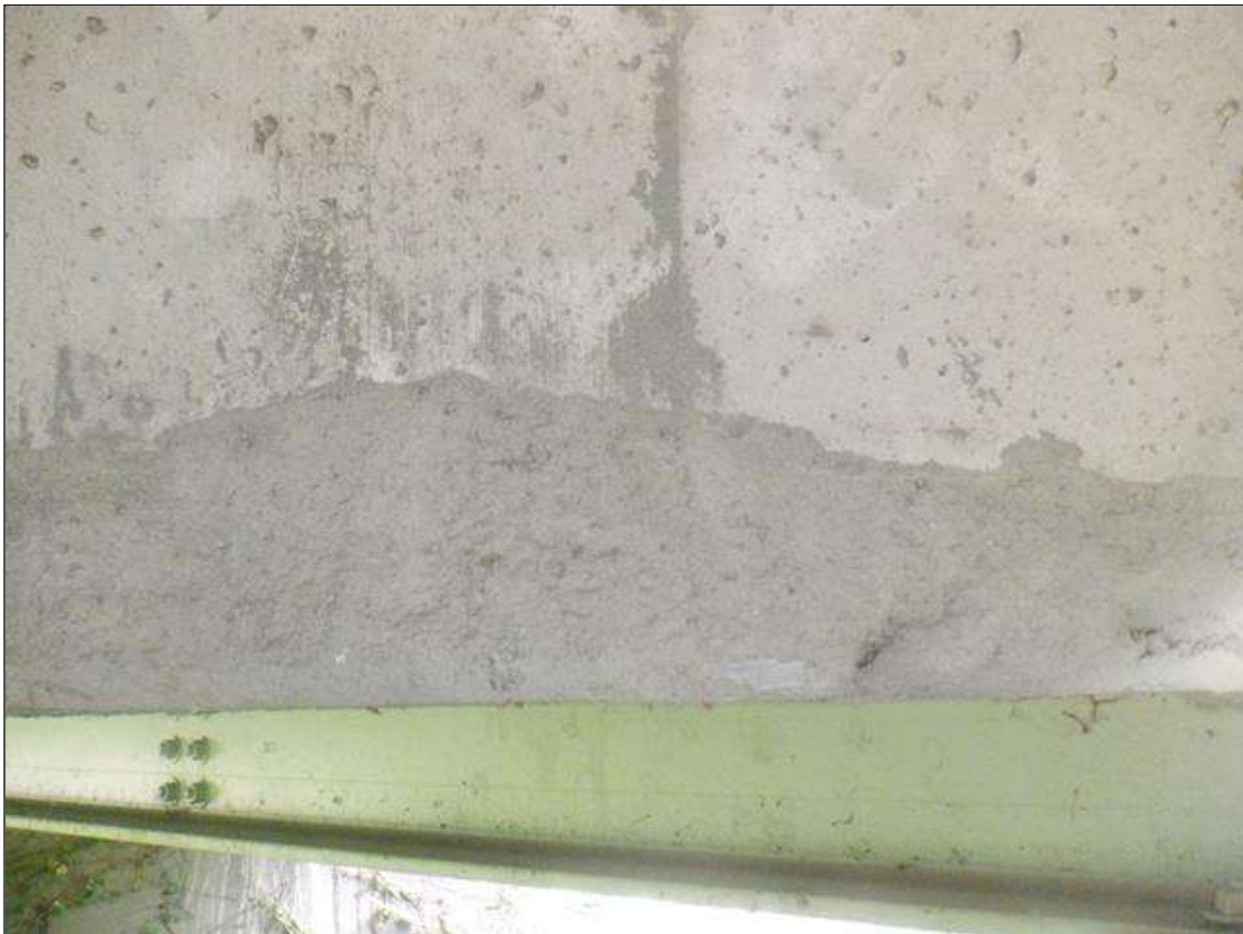
Span 7 Deck: 20 IN WIDE X 18 IN HIGH SOUND CONCRETE PATCHED AREA, BAY 1 END DIAPHRAGM, OVER BENT 7, NEXT TO BEAM 2.
