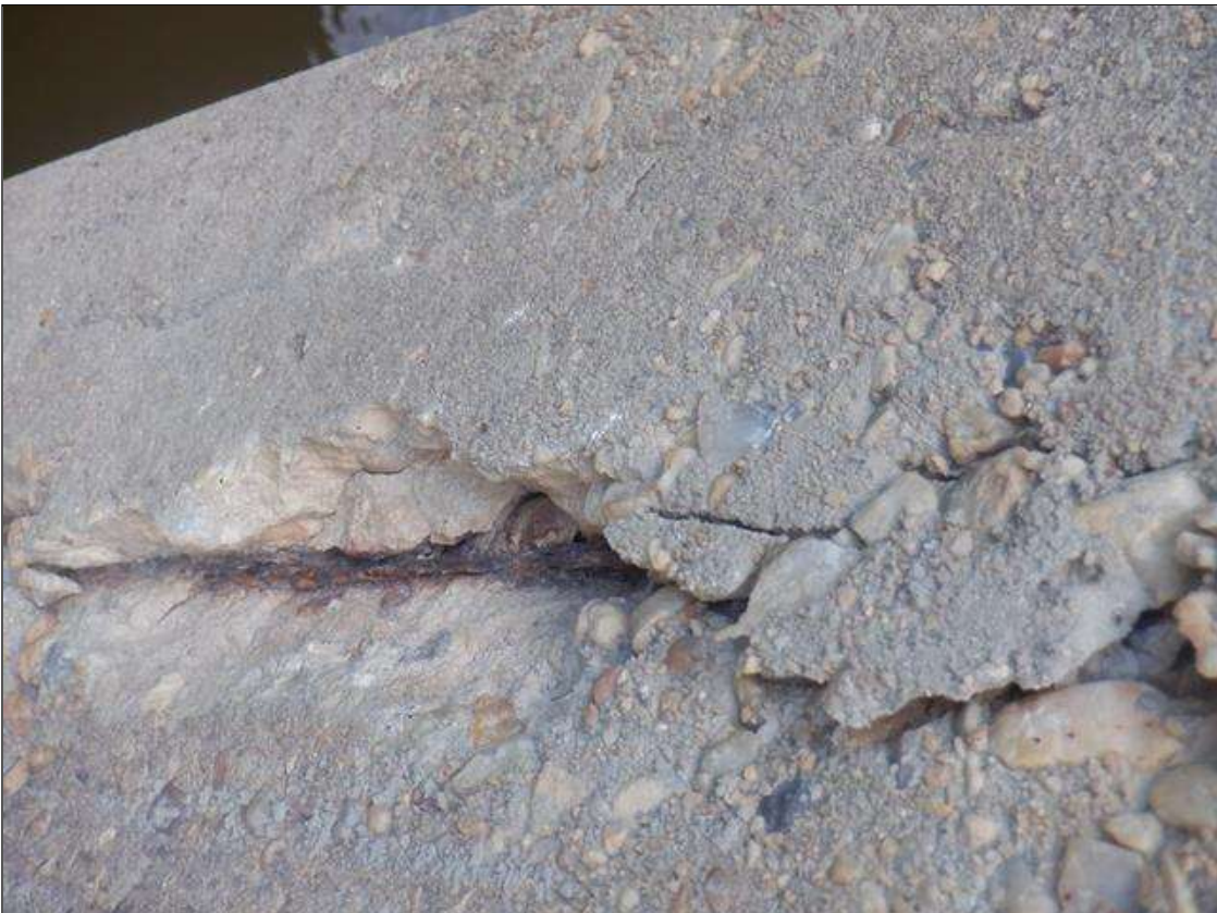
Bent 3 Pile 7: 4 FT HIGH X 4 IN WIDE SPALL 5 FT FROM WATER LEVEL, WITH EXPOSED REINFORCEMENT IN EAST FACE. 90% SECTION REMAINING IN EXPOSED REINFORCEMENT (PAR).
