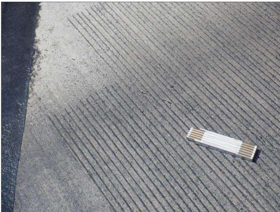
Span 8 Wearing Surface: UP TO 0.05 IN WIDE X 8 FT LONG DIAGONAL CRACKS EXTENDING FROM EXPANSION JOINT AT END BENT 2
