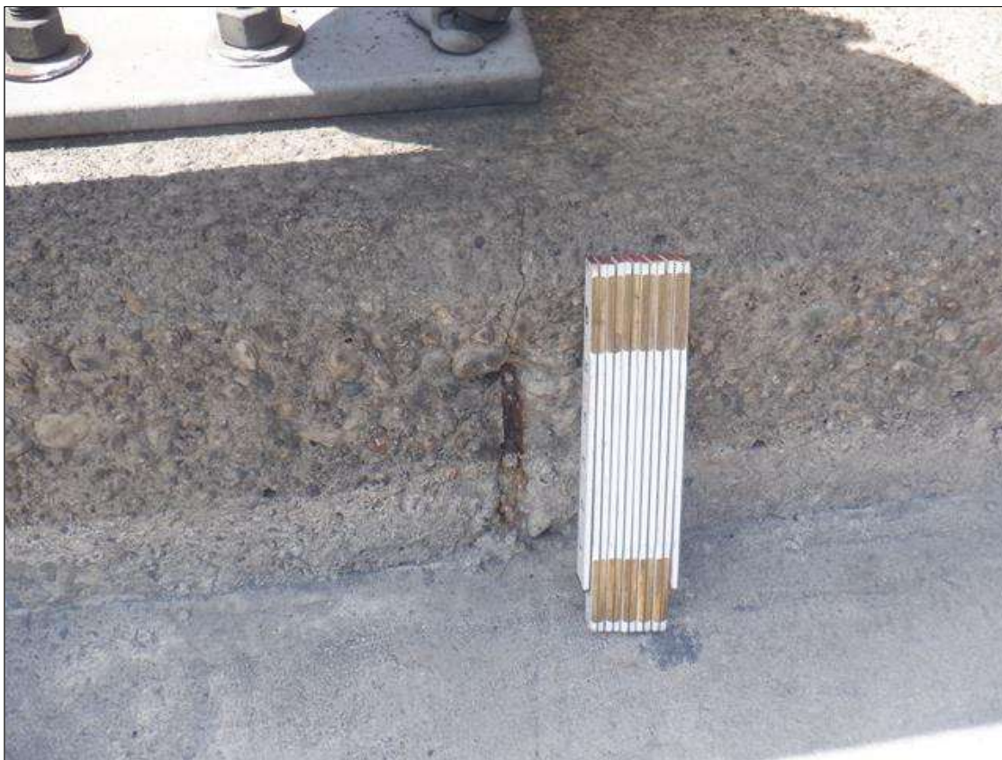
Span 3 Left Bridge Rail: TWO (2) SPALLS UP TO 8 IN IN DIAMETER X 1 IN DEEP WITH EXPOSED REINFORCEMENT IN BOTTOM OF CURB AT 6 FT AND 10 FT FROM BENT 3 JOINT. NO MEASUREABLE SECTION LOSS IN EXPOSED REINFORCEMENT.
