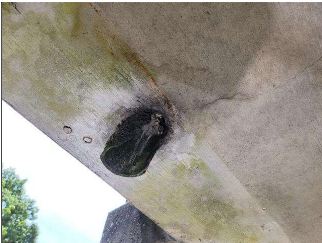
SEVERAL BROKEN DRAINAGE PIPES UNDER BOTH OVERHANGS
