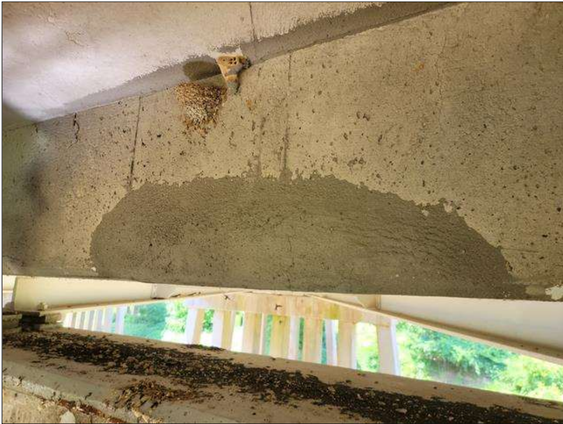
Span 6 Deck: 28 IN LONG X 1 FT HIGH SOUND CONCRETE PATCH IN BAY 2 END DIAPHRAGM, AT BENT 5. PATCH EXHIBITS HAIRLINE VERTICAL CRACKING, SCATTERED.
