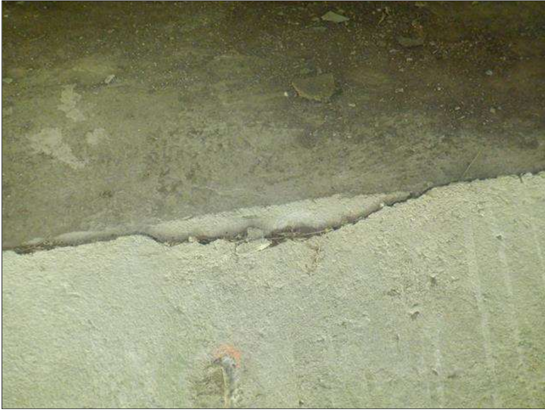
UP TO 12 IN LONG X 1/8 IN WIDE HORIZONTAL CRACK IN TOP OF BERM IN SLOPE PROTECTION AT END BENT 1
