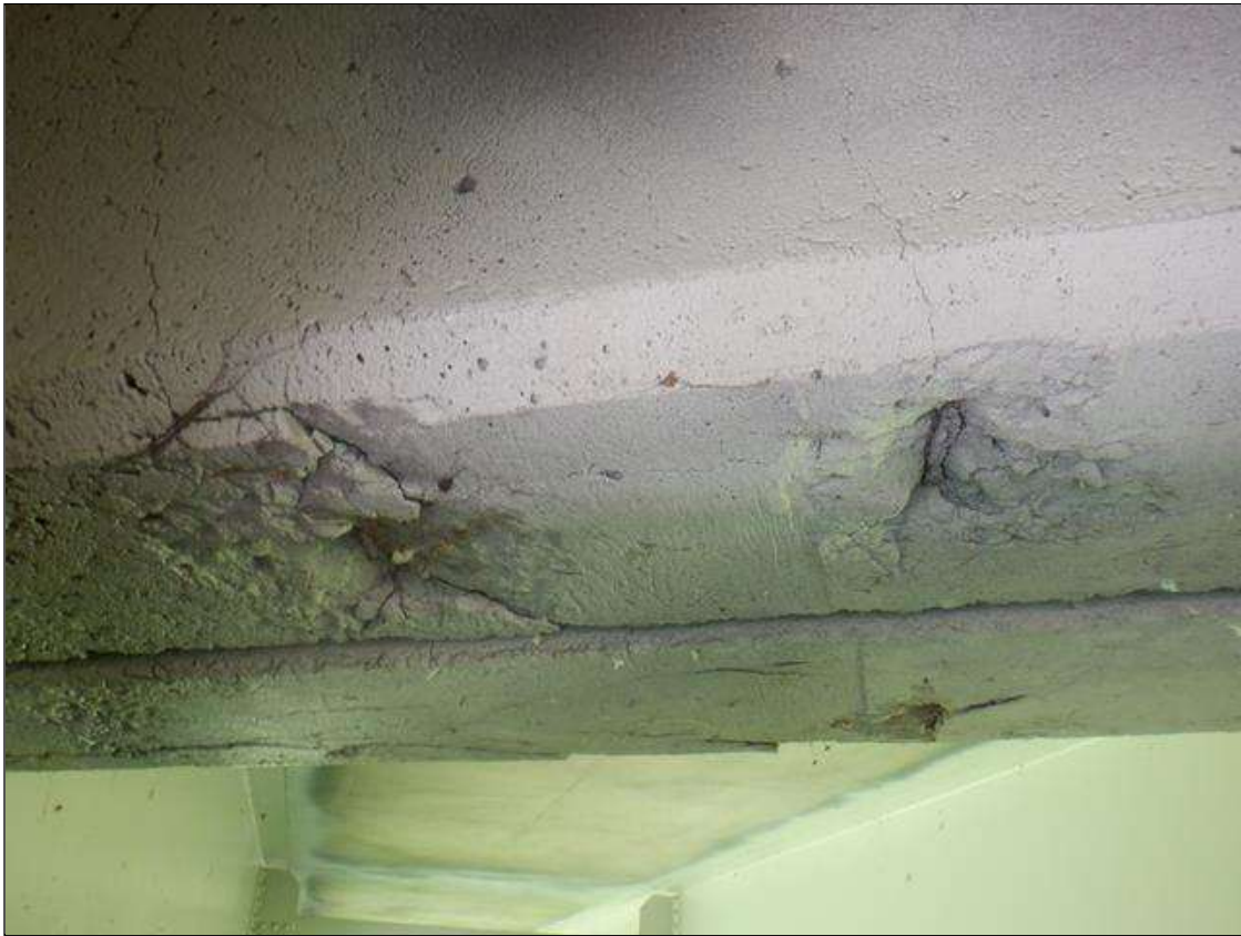
Span 1 Deck: (2) 6 IN DIAMETER X 3/4 IN DEEP SPALLS, UNDERSIDE OF BAY 1 END DIAPHRAGM, AT BENT 1.
