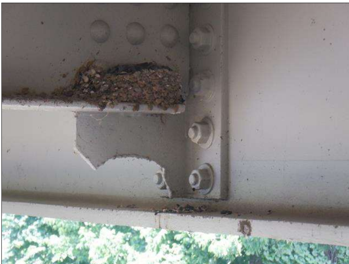
Span 4 Beam 1: UP TO 2 IN HIGH OF SECTION CUT OUT AT BOTTOM OF INTERMEDIATE STIFFENER. PAR IS NOT ISSUED AS IT APPEARS TO BE FROM A BRIDGE REPAIR
