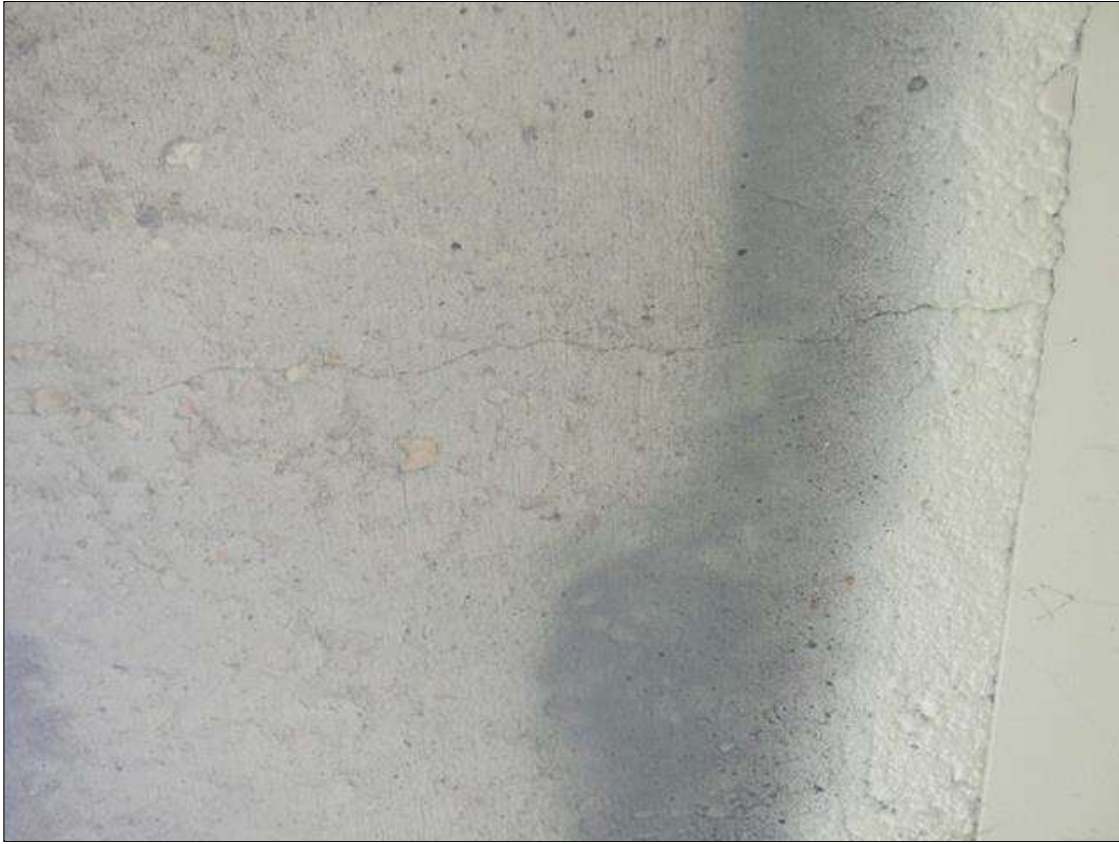
Span 7 Deck: EIGHT (8) UP TO 0.03 IN WIDE X UP TO 3 FT LONG TRANSVERSE CRACKS IN LEFT OVERHANG. RIGHT OVERHANG TYPICAL.
