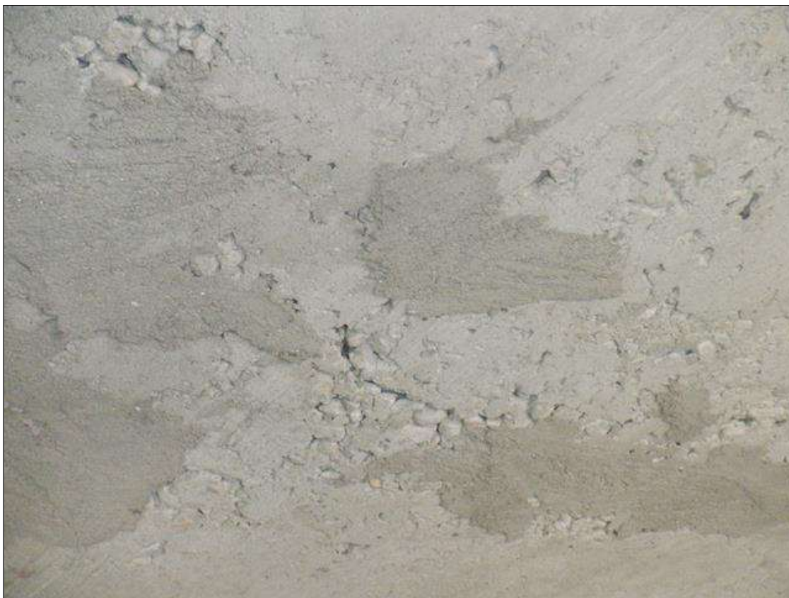
Span 7 Deck: SCATTERED AREAS OF HONEYCOMBING IN DECK UNDERSIDE IN ALL BAYS
