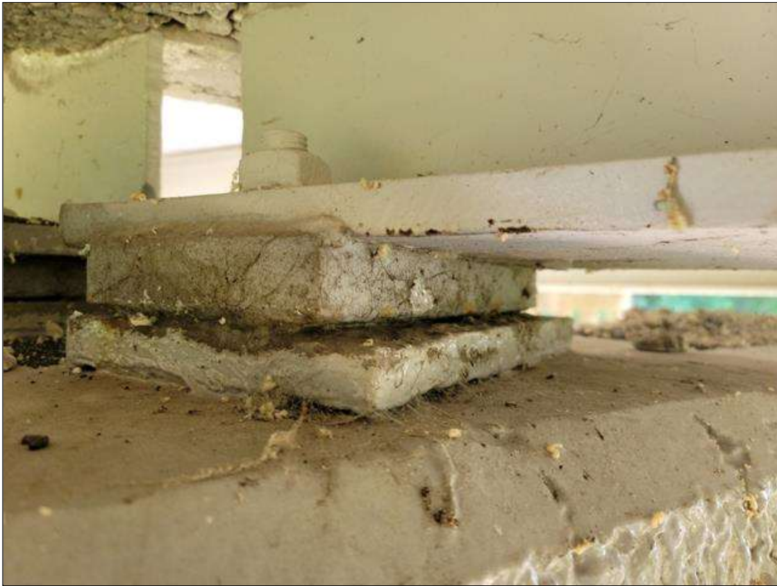
Span 5 Far Bearing: BEARINGS HAVE BEEN PAINTED SINCE PREVIOUS INSPECTION. SECTION LOSS REMAINS BENEATH THE PAINTED SURFACES. UP TO 90% SECTION REMAINING IN BOTH MASONRY AND SOLE PLATES.
