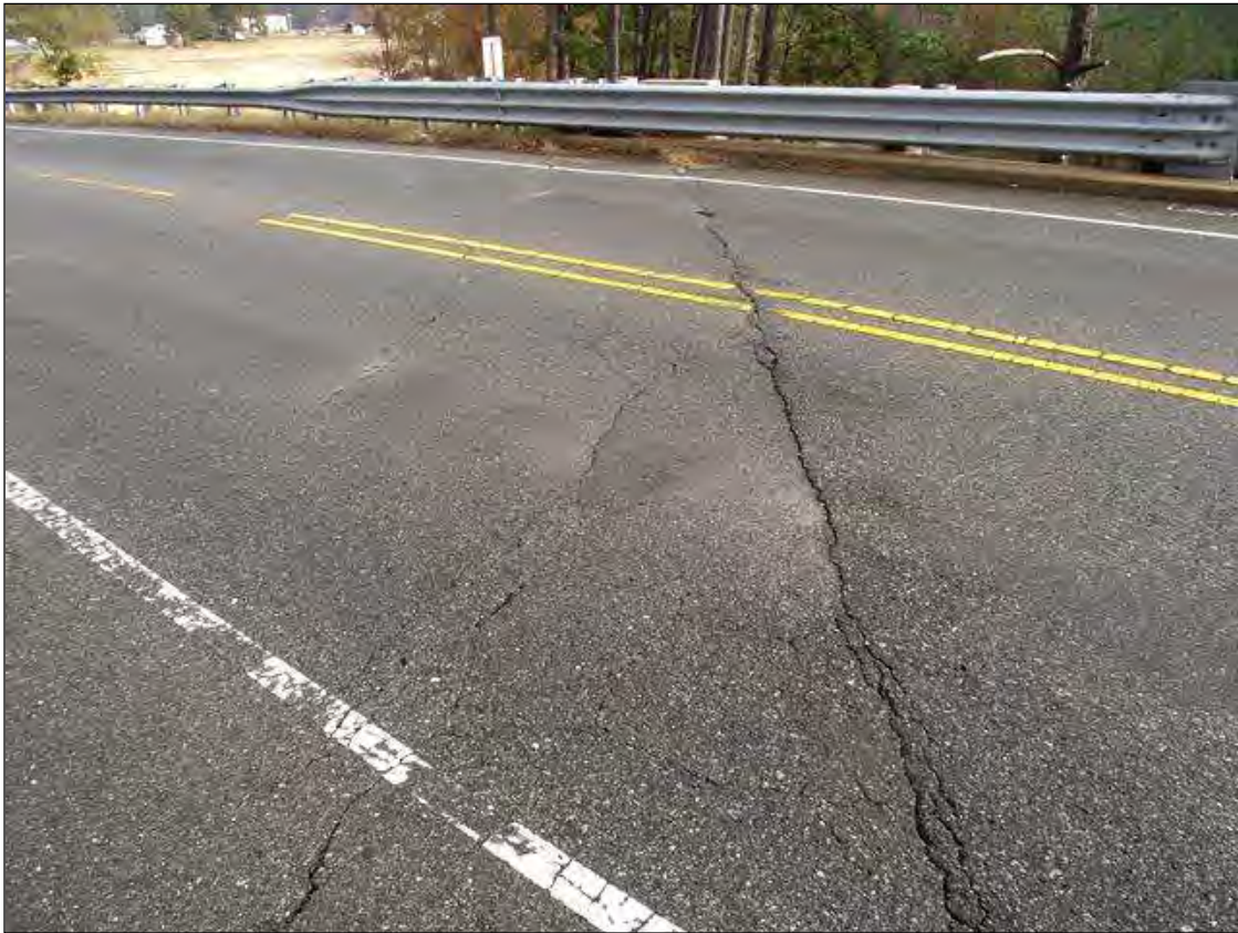
WEARING SURFACE CRACKED OVER END BENT 2 AND APPROACH 2
