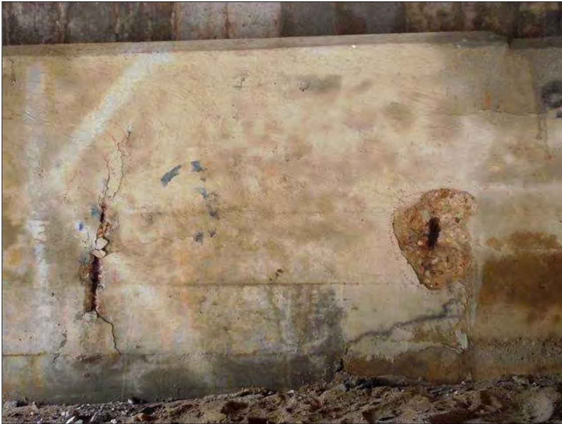
SPALLING WITH EXPOSED REBAR IN FACE OF CAP AT END BENT 1 BAY 4
