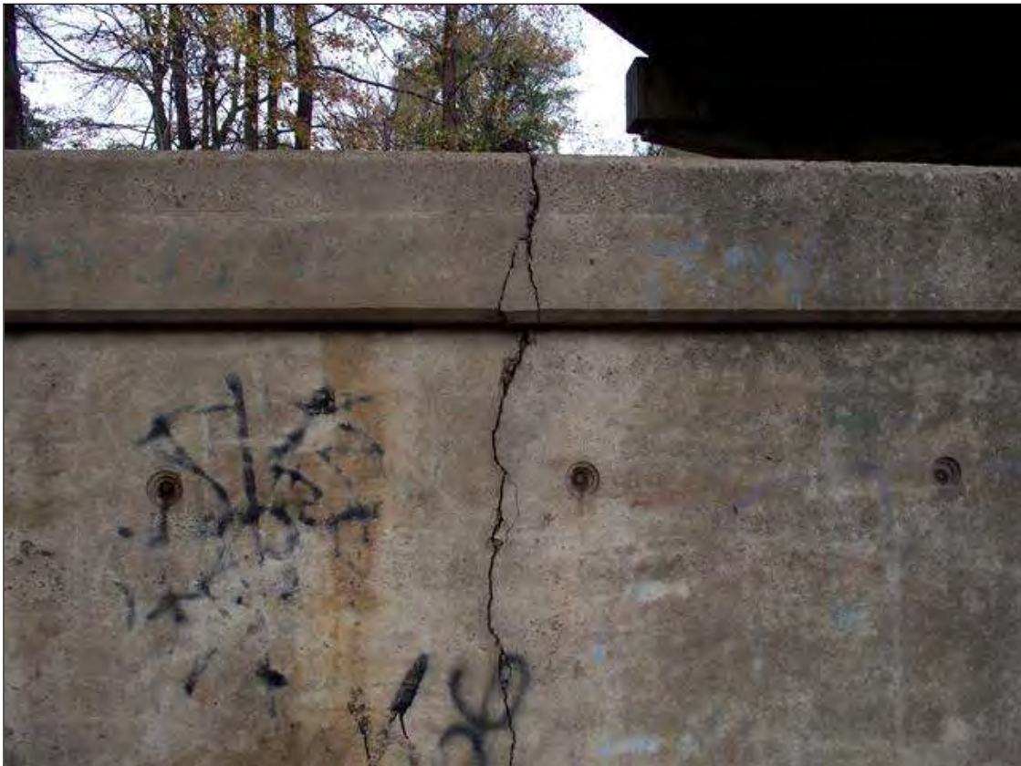
VERTICAL CRACK IN BENT 2 PEDESTAL SPAN 2 SIDE - EXTENDS OVER TOP AND DOWN SPAN 3 SIDE
