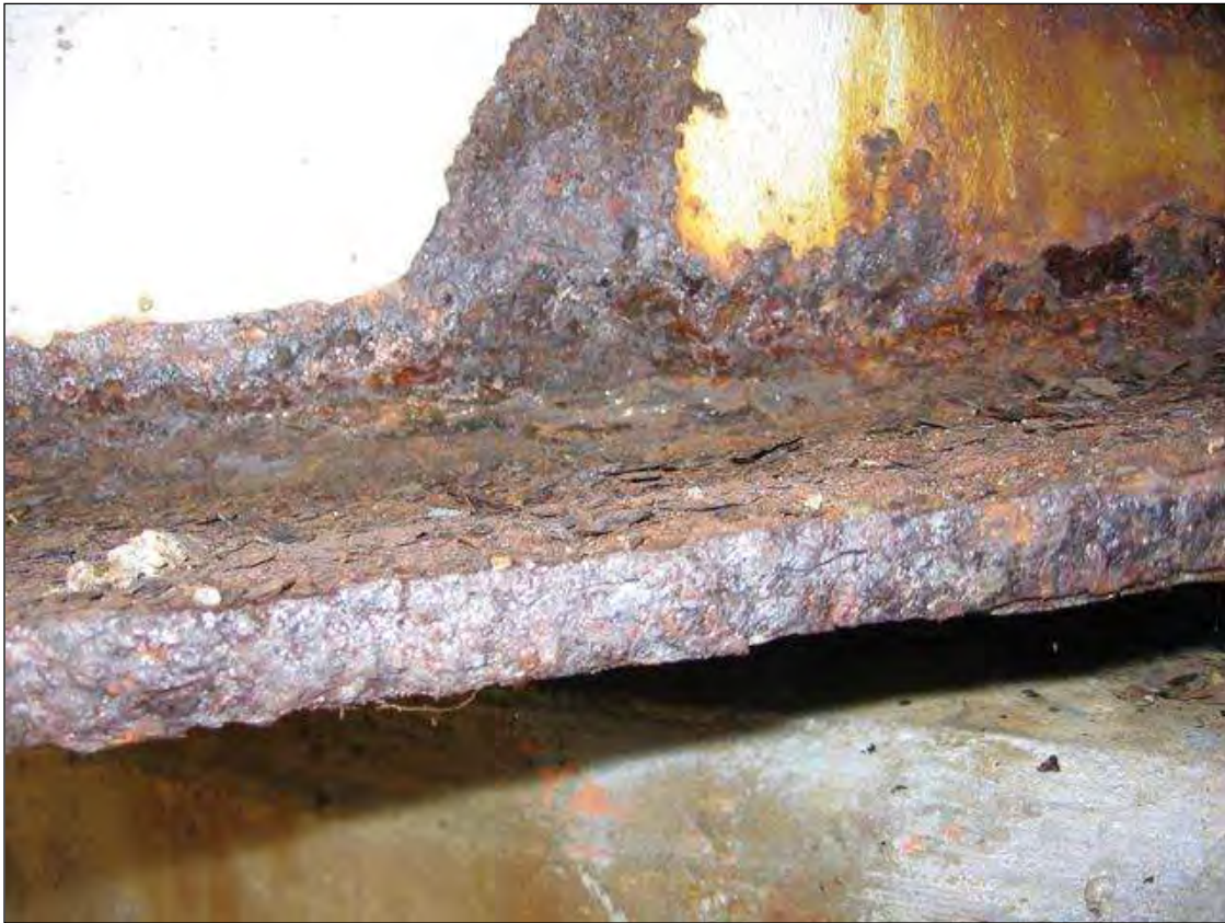
SECTION LOSS IN THE WEB AND BOTTOM FLANGE OF BEAM 5 IN SPAN 5 OVER BENT 4
