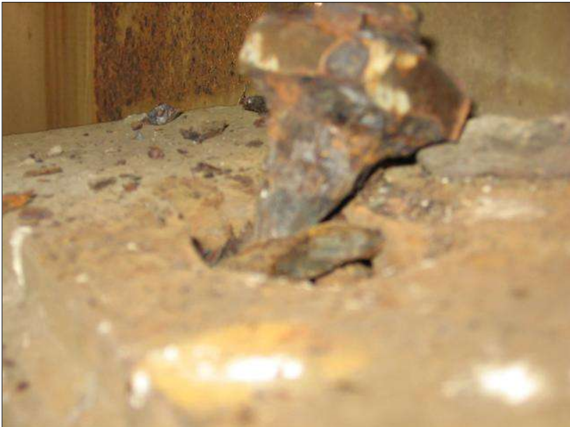
SECTION LOSS IN THE RIGHT SIDE ANCHOR BOLT FOR BEAM 4 IN SPAN 4 OVER BENT 3 - PRIORITY MAINTENANCE ISSUED
