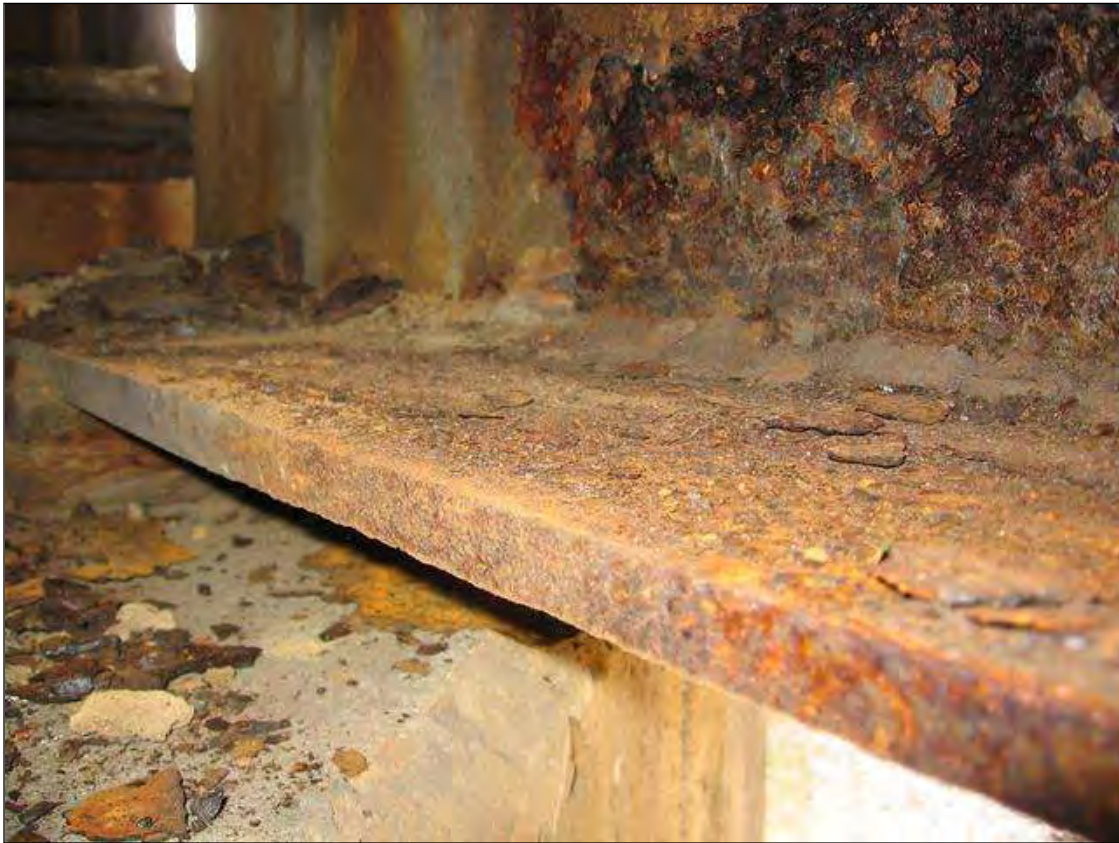
SECTION LOSS IN THE BOTTOM FLANGE OF BEAM 1 IN SPAN 3 OVER BENT 2
