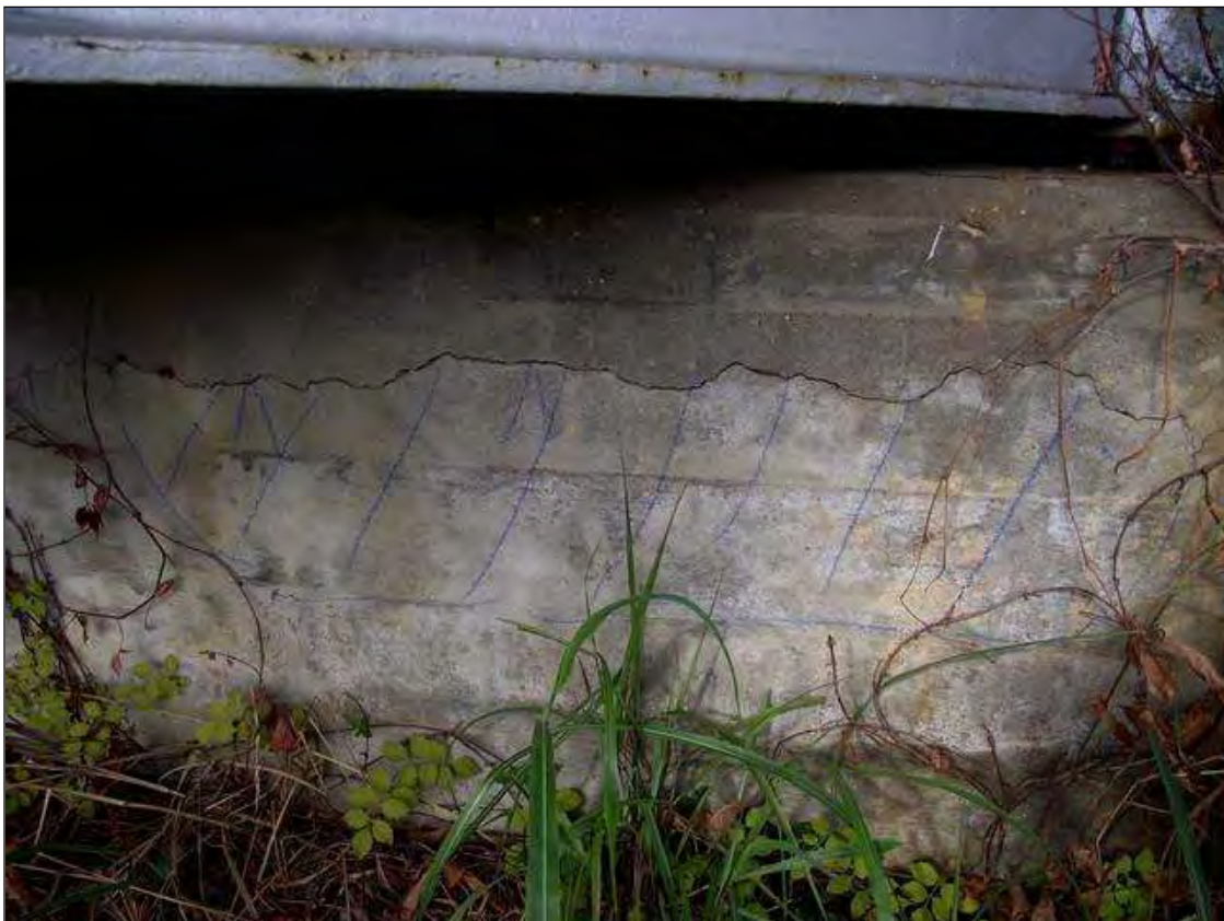
AREA OF DELAMINATION IN FACE OF CAP AT END BENT 2 UNDER BEAM 5
