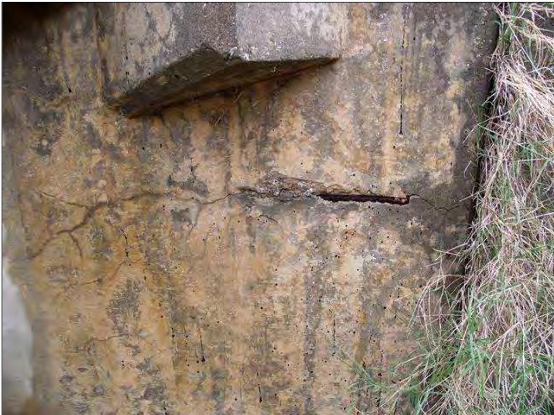
SPALLING WITH EXPOSED REBAR IN THE LEFT EXTERIOR BACKWALL AT END BENT 1
