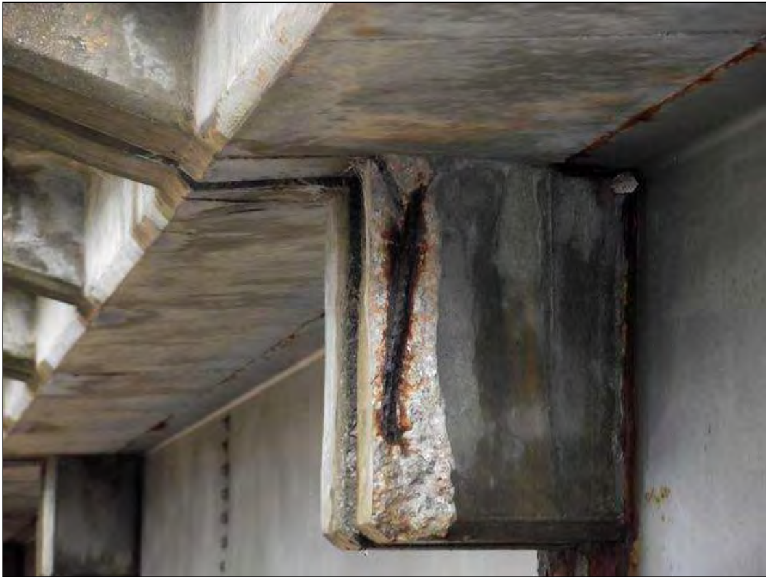
LEFT EXTERIOR END DIAPHRAGM IN SPAN 1 AT BENT 1 SPALLED WITH SECTION LOSS TO EXPOSED REBAR
