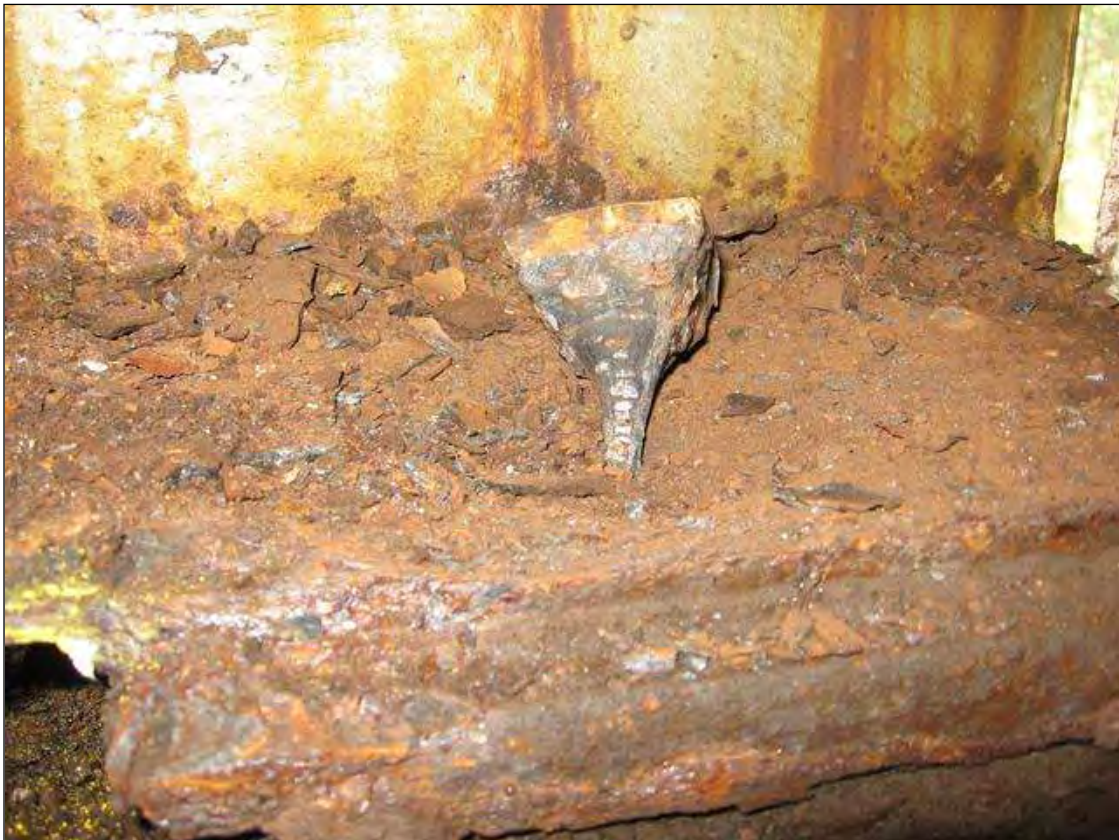
SECTION LOSS IN THE LEFTSIDE ANCHOR BOLT FOR BEAM 5 IN SPAN 4 AT BENT 3 - PRIORITY MAINTENANCE ISSUED
