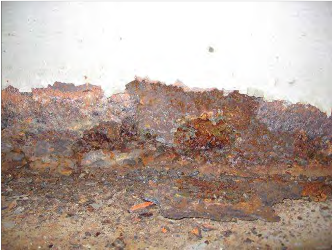
SECTION LOSS IN THE WEB OF BEAM 1 IN SPAN 1 OVER BENT 1
