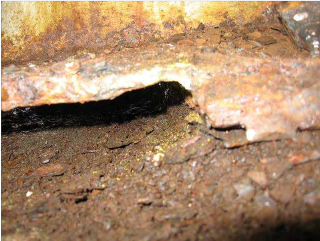
SECTION LOSS IN THE BOTTOM FLANGE OF BEAM 5 IN SPAN 4 OVER BENT 3
