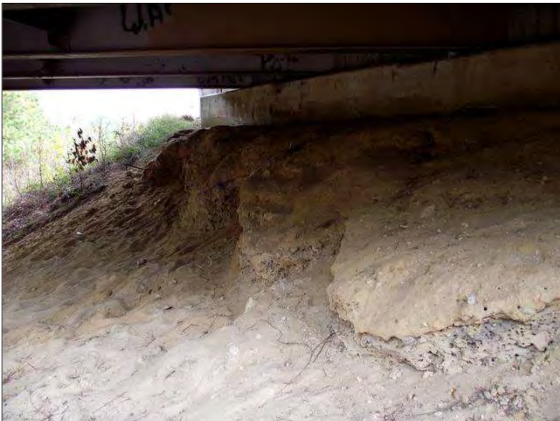
EROSION AT TOP OF SLOPE UNDER SPAN 1
