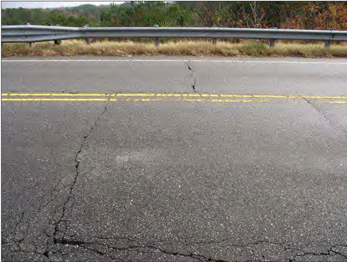
LONGITUDINAL AND TRANSVERSE CRACKS IN APPROACH 1
