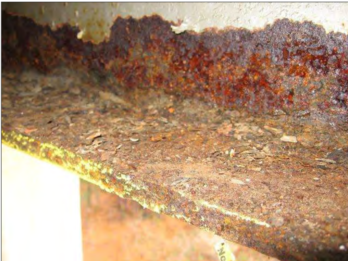
SECTION LOSS IN THE WEB AND BOTTOM FLANGE OF BEAM 5 IN SPAN 1 OVER BENT 1
