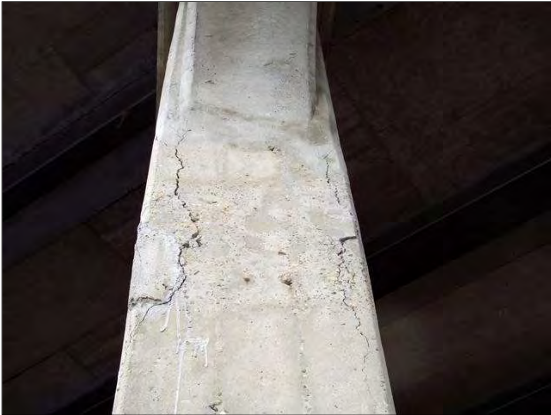
CRACKING AND DELAMINATION IN THE RIGHT SIDE OF COLUMN 2 AT BENT 3 AND SPAN 4 SIDE
