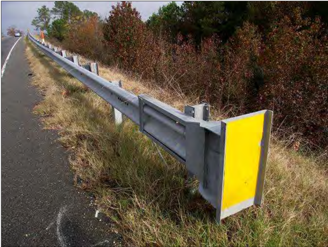
RIGHT SIDE GUARDRAIL TERMINAL END APPROACH 1
