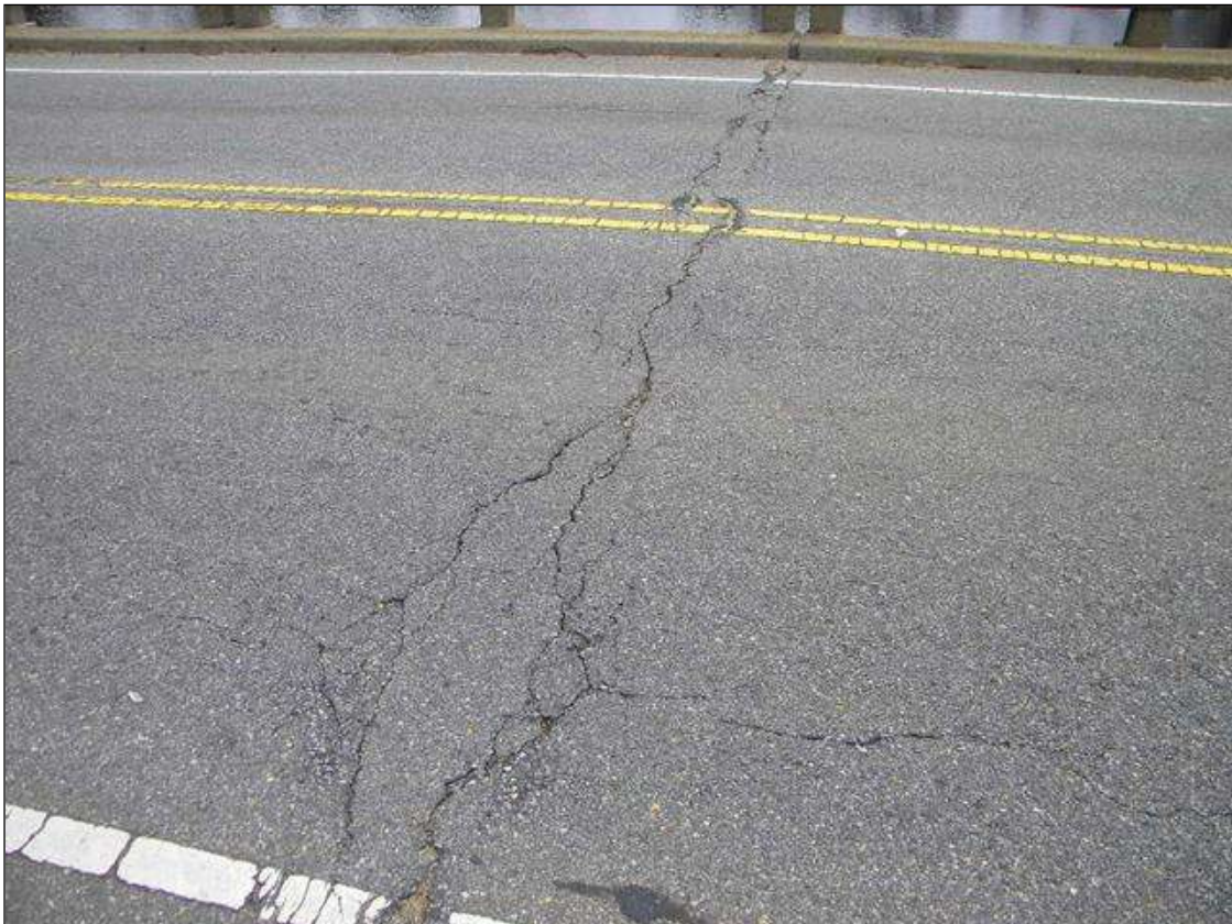
TRANSVERSE CRACKING AND SMALL VOIDS IN WEARING SURFACE OVER BENT 2
