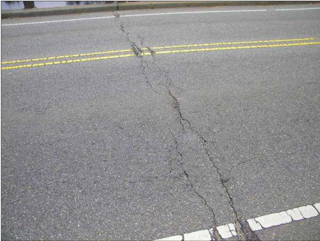
TRANSVERSE CRACKING IN WEARING SURFACE OVER BENT 3
