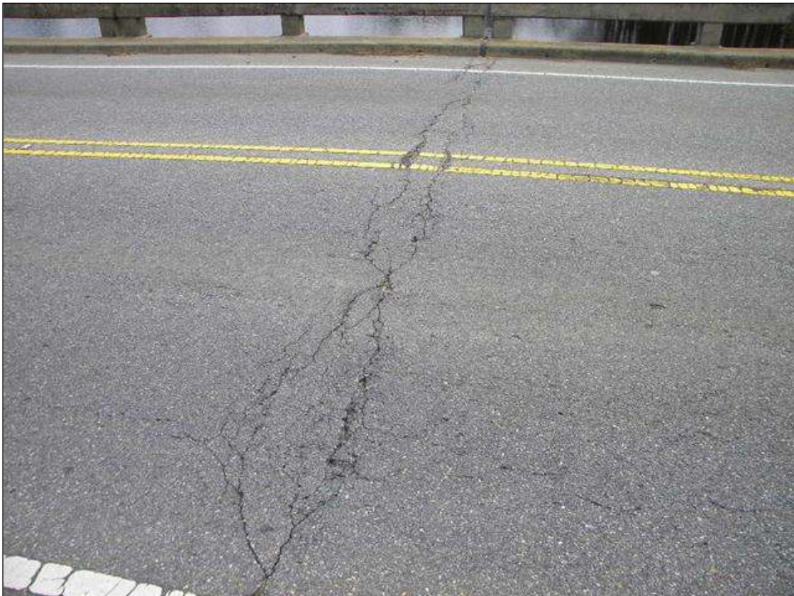
TRANSVERSE CRACKING IN WEARING SURFACE OVER BENT 1
