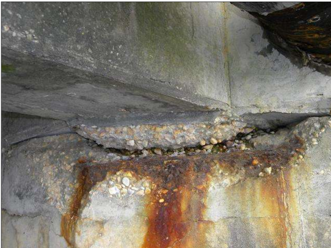
SPALLING UNDER GIRDER 1 BEARING AT ABUTMENT 1
