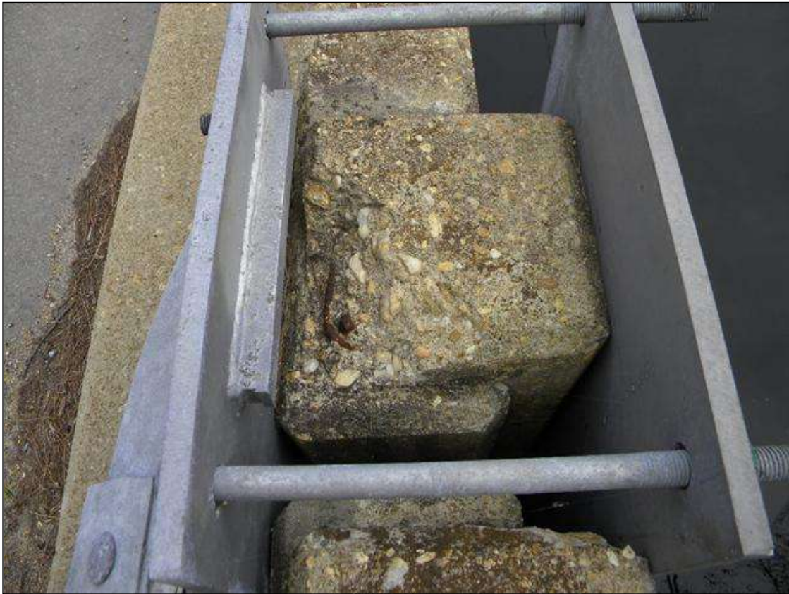
RIGHT SIDE GUARDRAIL POST AT GUARDRAIL CONNECTION IN SPAN 1 SPALLED
