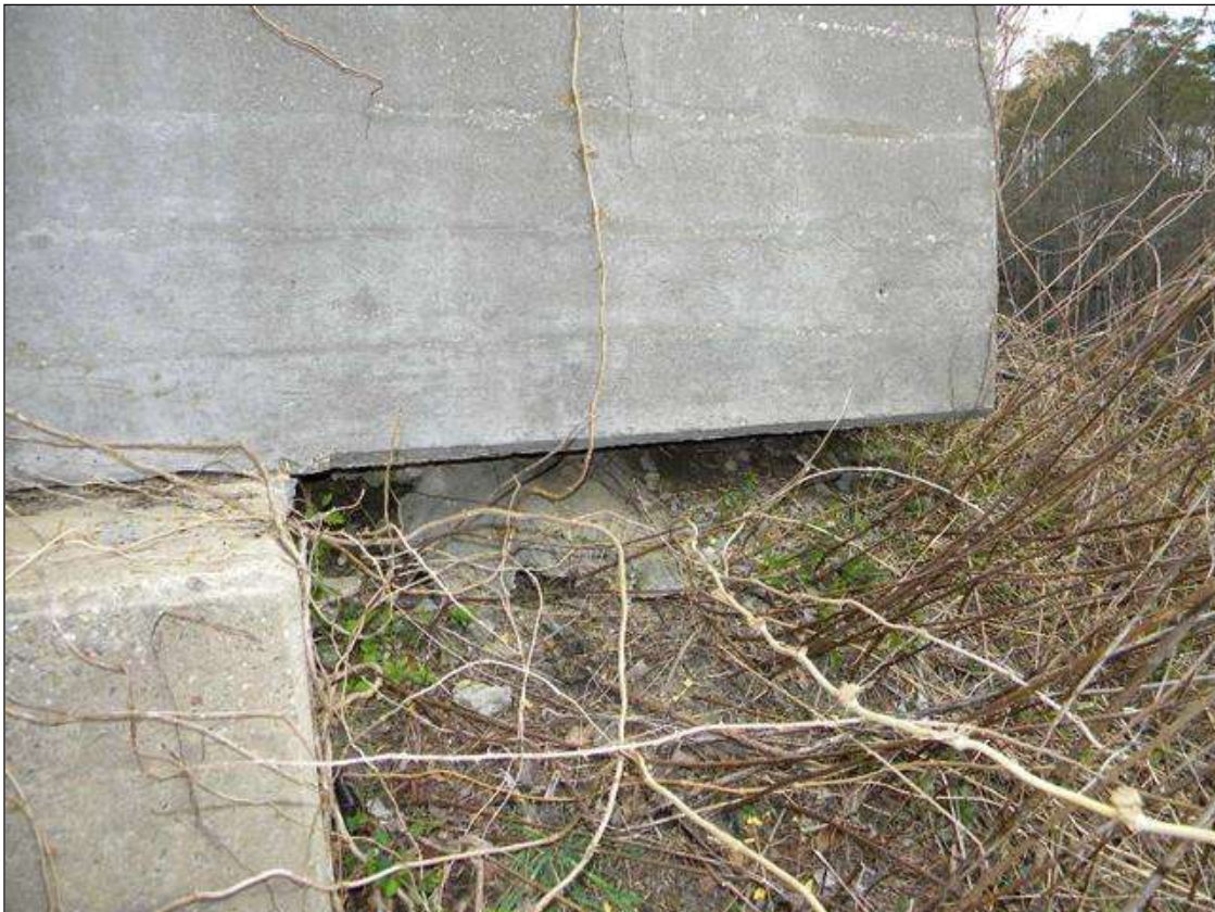
UNDERMINING AT END BENT 2 RIGHT SIDE WINGWALL - LEFT SIDE SIMILAR
