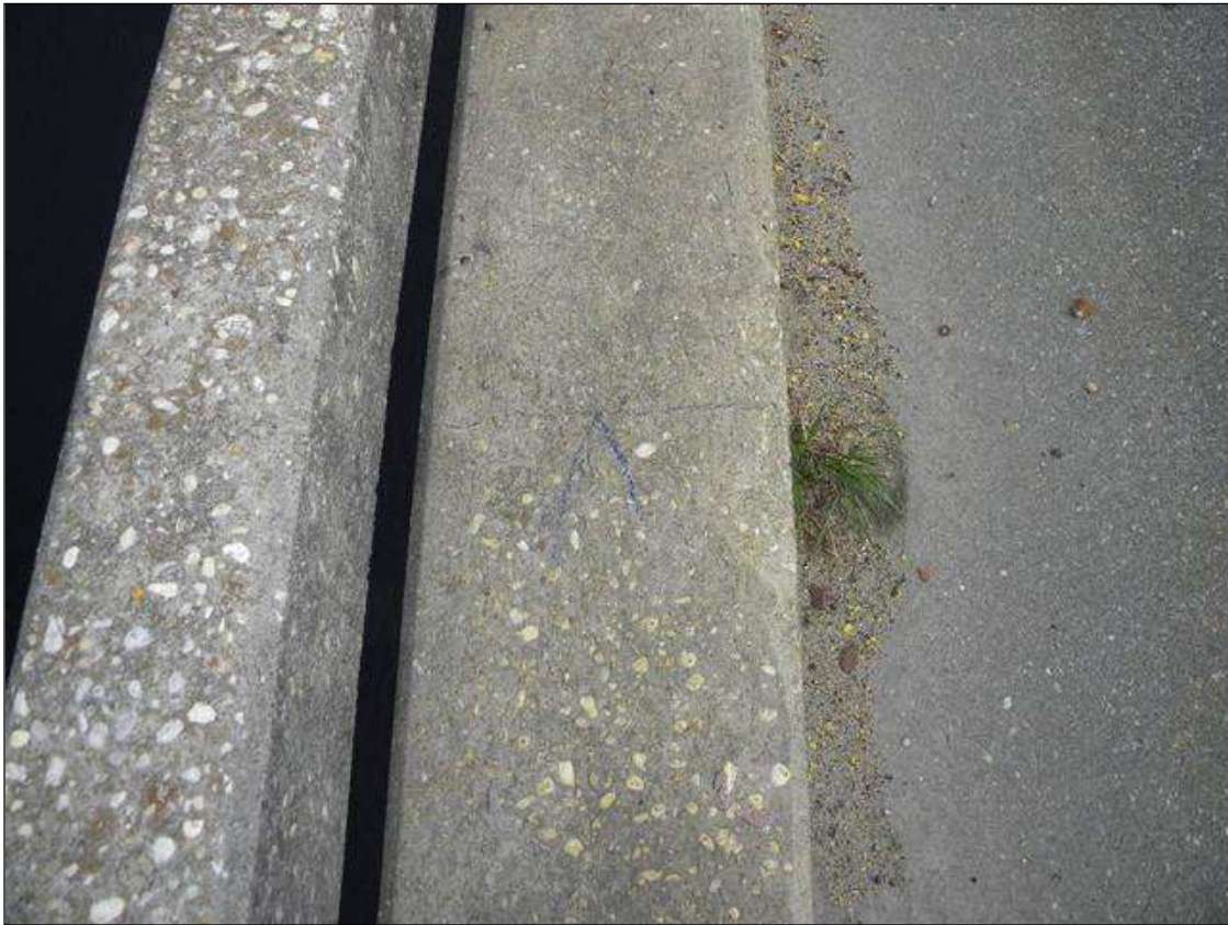
RANDOM TRANSVERSE CRACK IN TOP OF CURBLINES
