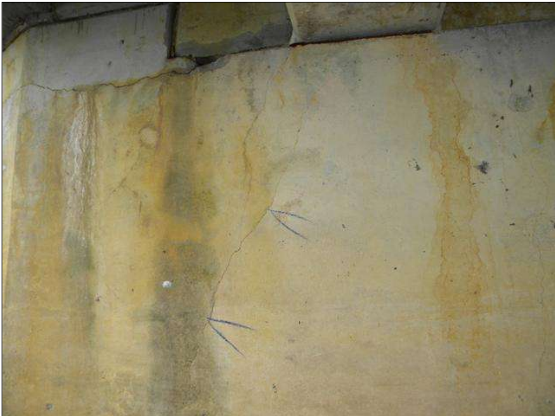
RANDOM VERTICAL CRACKS IN FACE OF ABUTMENT 1
