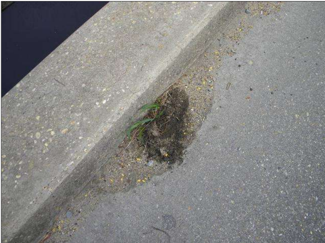
DECK DRAINS CLOGGED WITH VEGETATION
