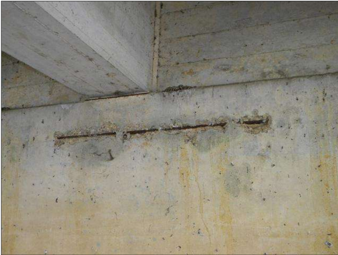
SPALL WITH EXPOSED REBAR IN ABUTMENT 1 UNDER GIRDER 3
