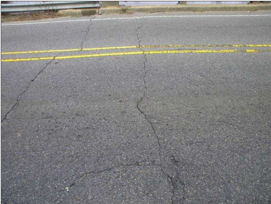
TRANSVERSE CRACK AND UNEVENNESS OVER END BENT 1 WEARING SURFACE
