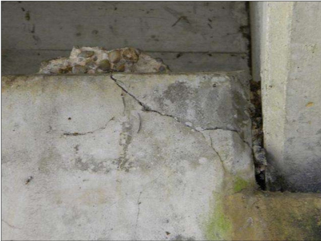
CRACK IN GIRDER 4 RETAINING BLOCK AT BENT 2 SPAN 3 SIDE
