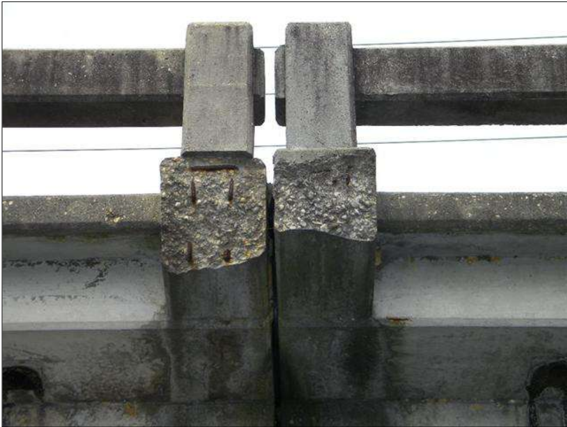
GUARDRAIL POST BASES AT THE RIGHT SIDE OF BENT 3 SPALLED WITH EXPOSED REBAR
