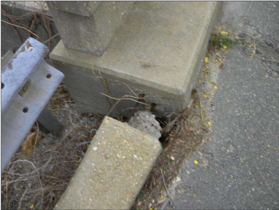
RIGHT SIDE CURB END TREATMENT AT END BENT 2 PULLED OUT AND SETTLED
