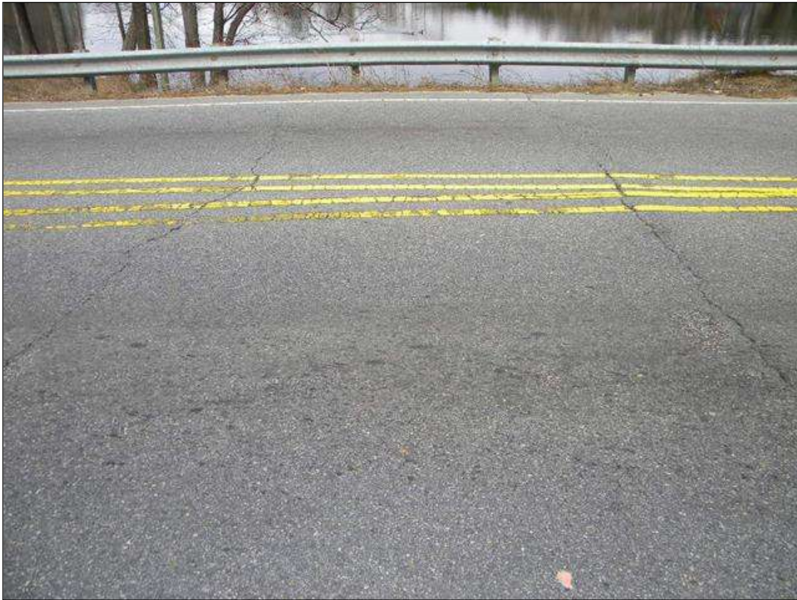
TRANSVERSE CRACKS IN APPROACH 1 WEARING SURFACE
