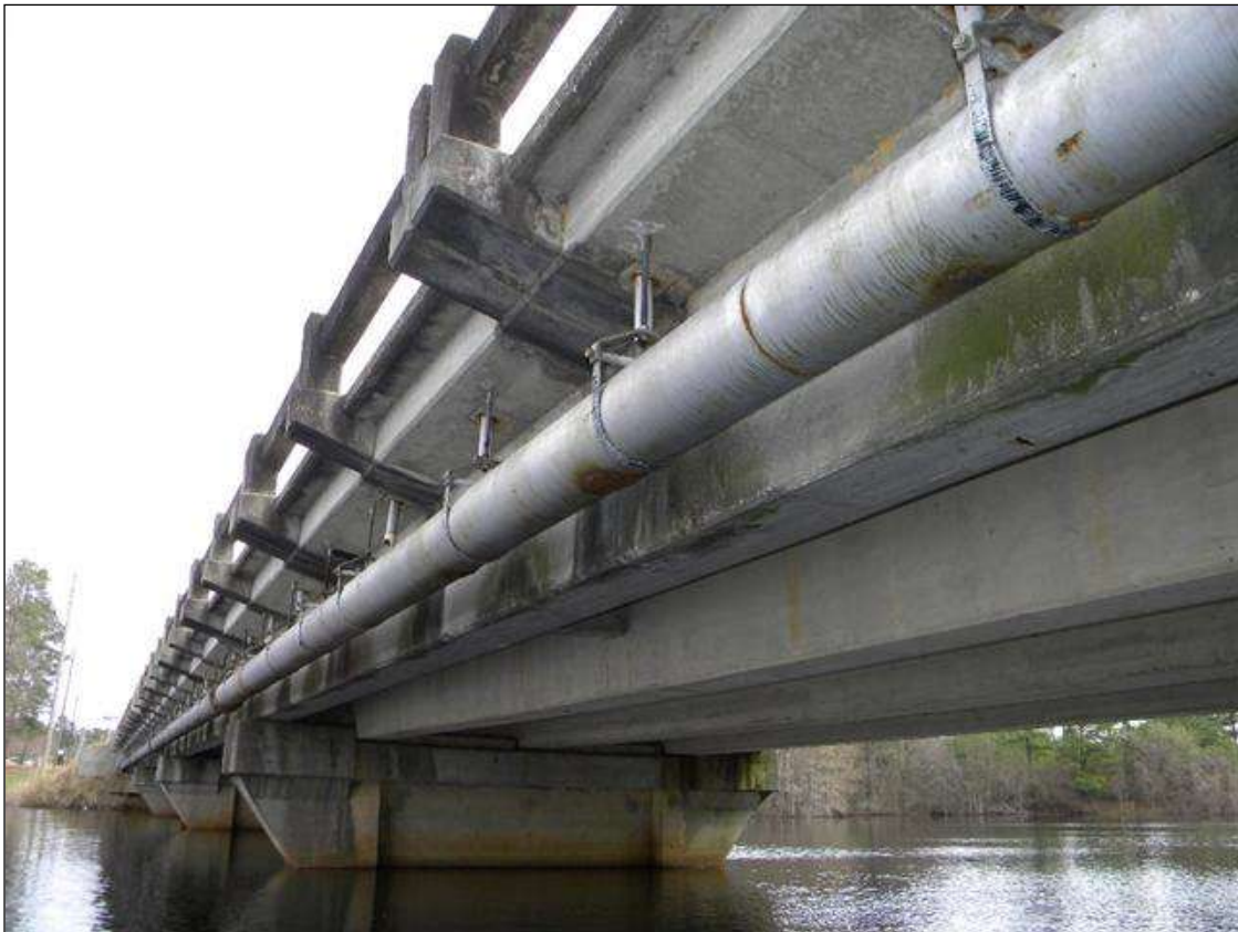
UTILITIES ALONG THE LEFT SIDE OVERHANG
