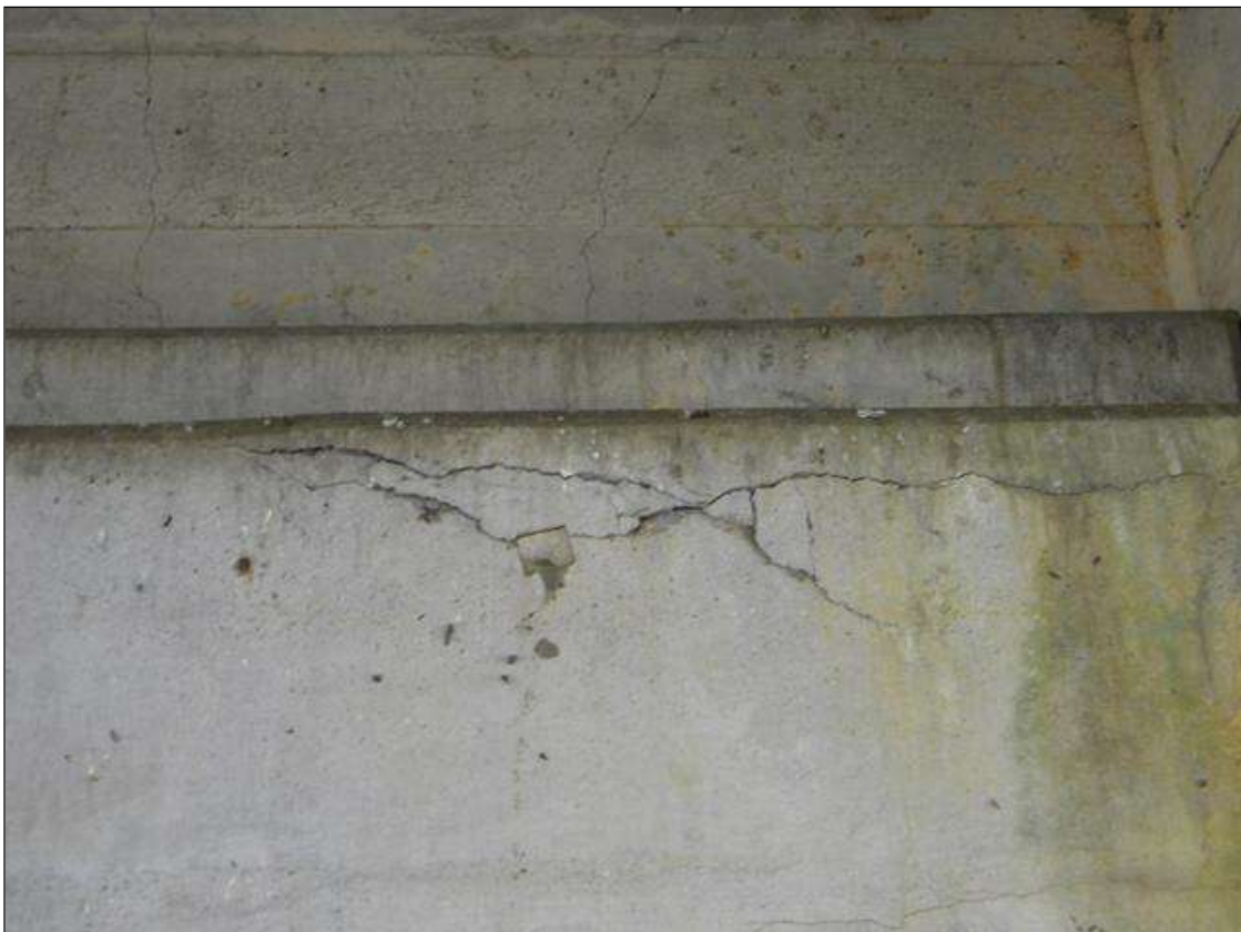
CRACKING IN FACE OF CAP AT BENT 3 BAY 3 SPAN 3 SIDE
