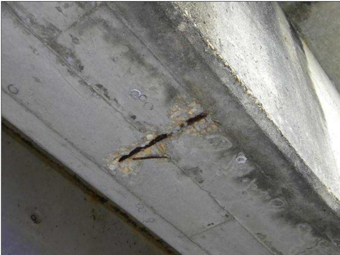
SHALLOW SPALLING WITH EXPOSED REBAR IN BOTTOM OF GIRDER 5 IN SPAN 2 AT 1/3 POINT FROM BENT 1
