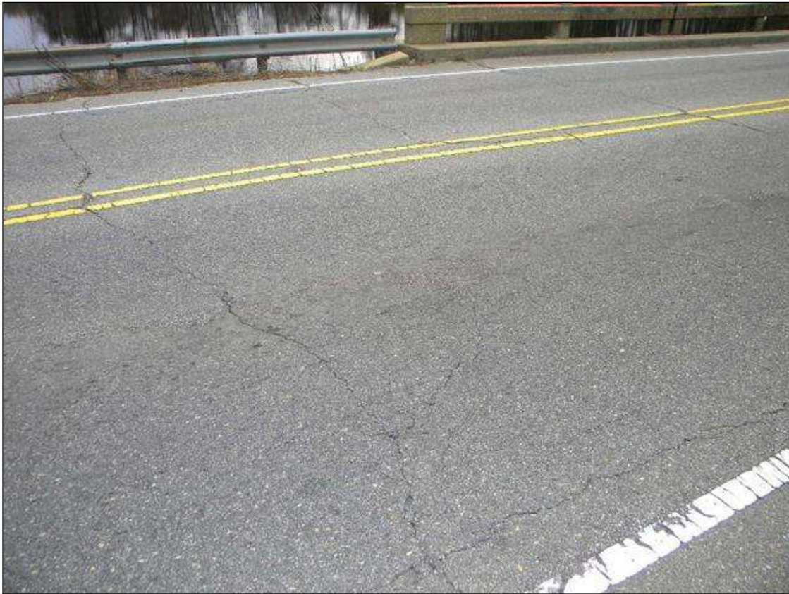
TRANSVERSE AND LONGITUDINAL CRACKS IN APPROACH 2 WEARING SURFACE
