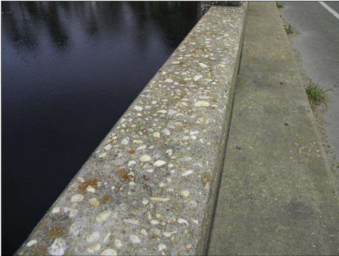
GUARDRAILS SCALED WITH COARSE AGGREGATE EXPOSED
