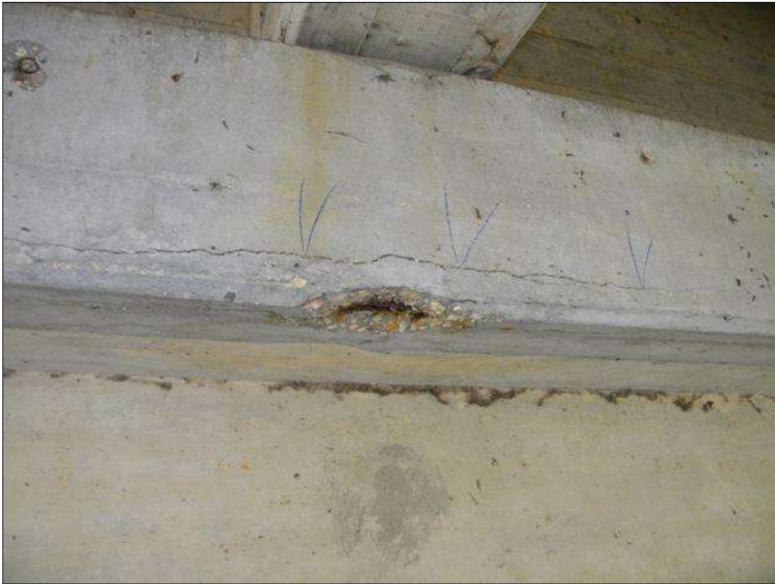
SPALLING AND DELAMINATION IN BOTTOM EDGE OF BENT 1 CAP SPAN 1 SIDE
