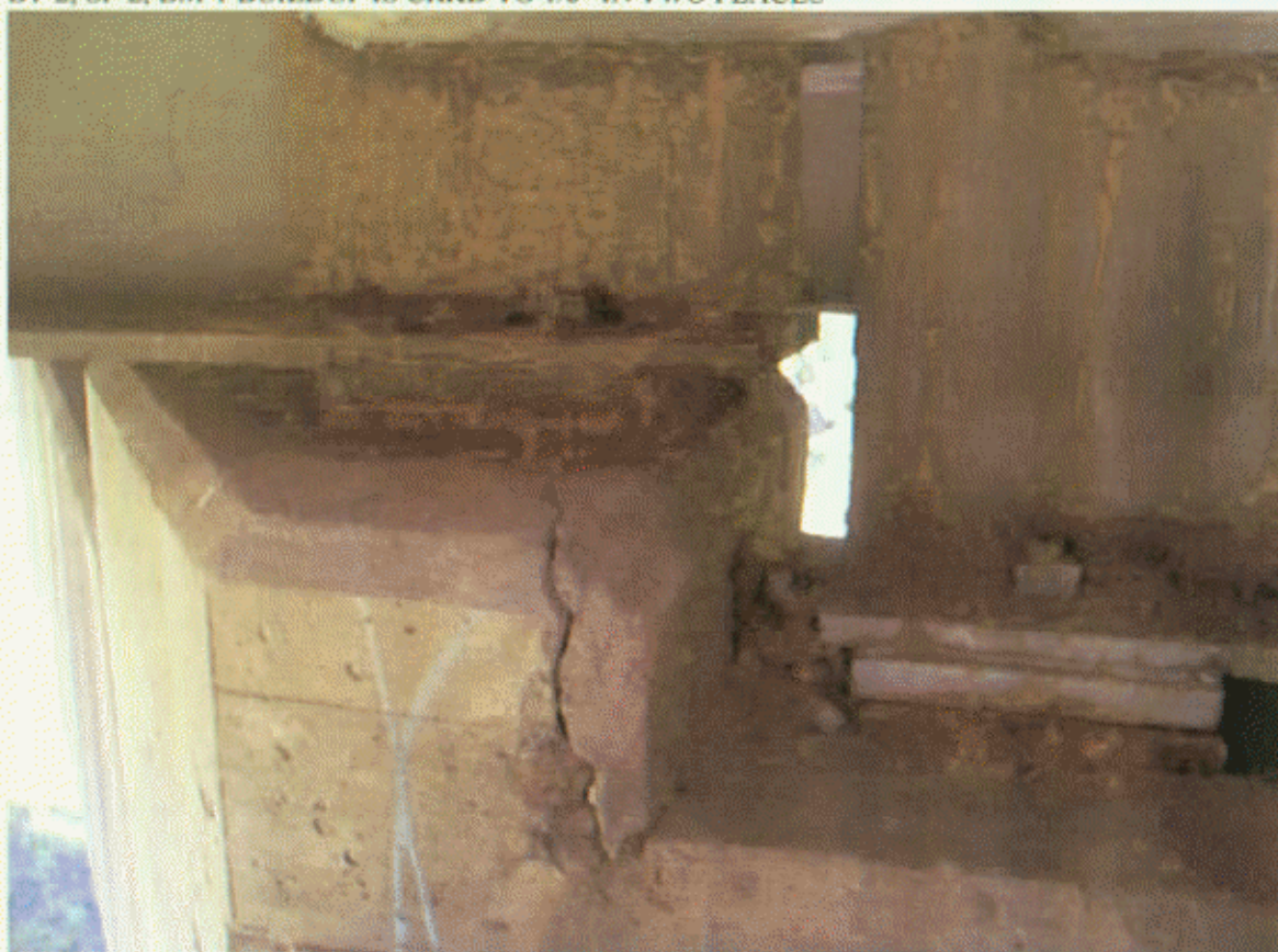
BT-2, SP-2; BM-3 HAS CRK TO 3/16" IN BUILDUP ON RT SIDE
