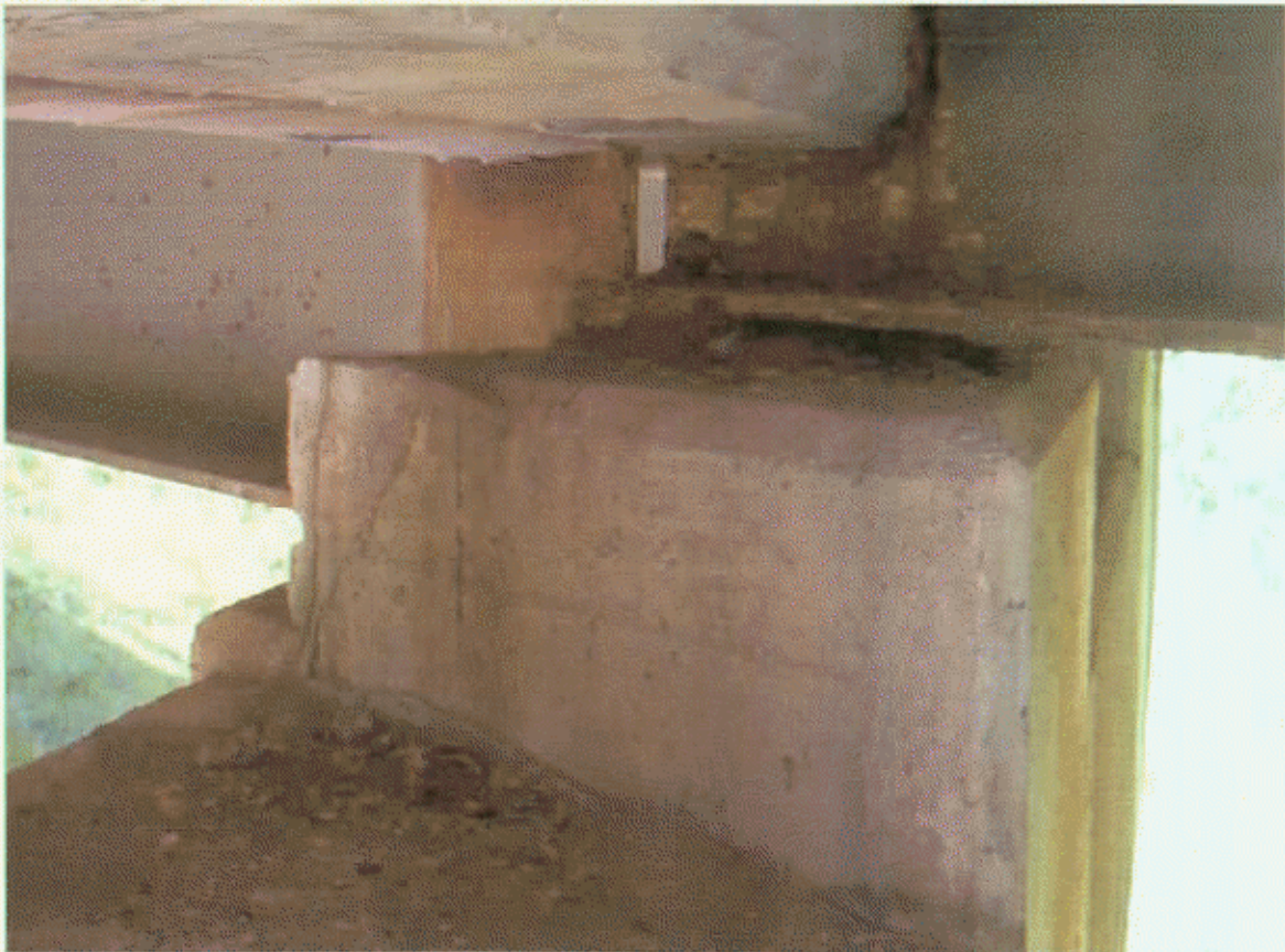
BT-3, SP-4; BUILDUP IS CRKD TO 1/32" UNDER BM-3 AND RT ANCHOR BOLT IS HEAVILY RUSTED
