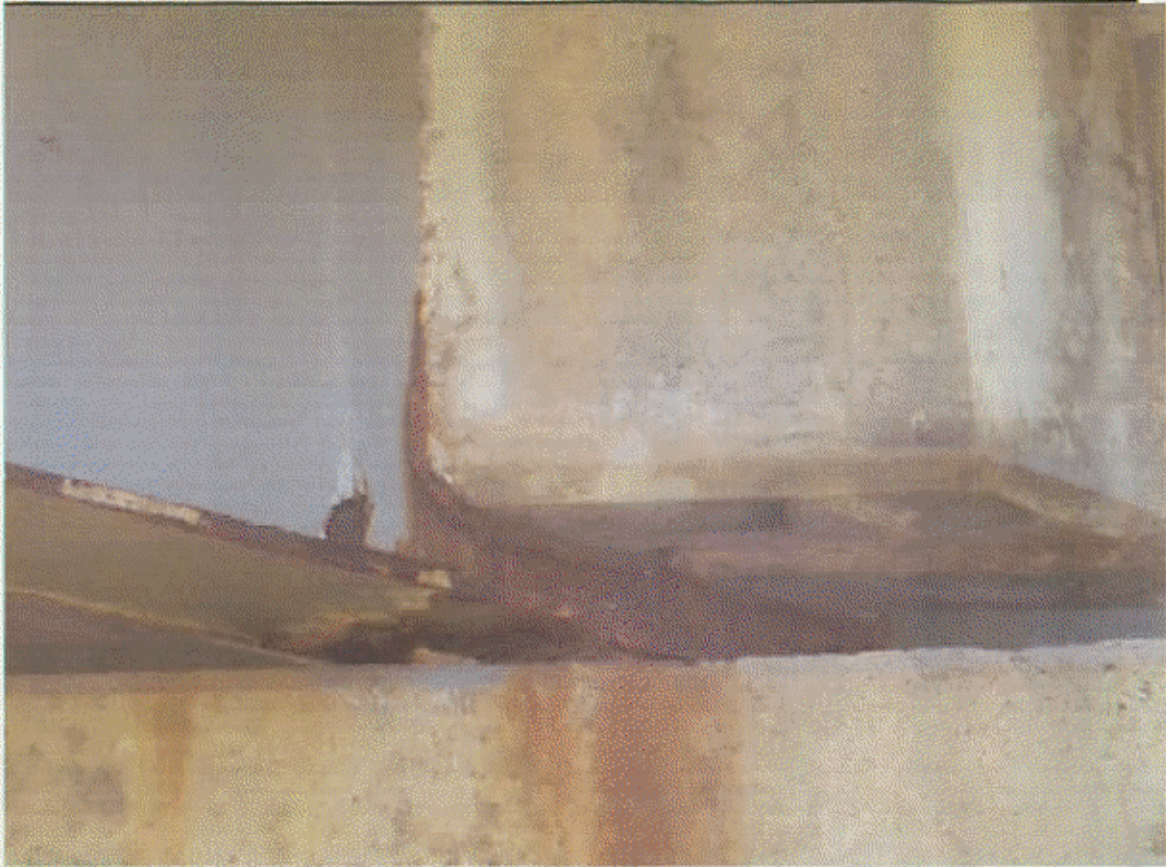
BT-4, SP-5; BEARING AT BM-5 IS HEAVILY RUSTED
