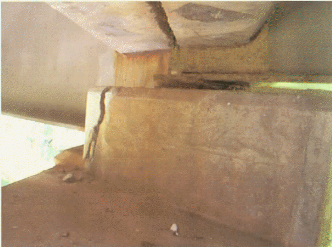
BT-3, SP-4; BUILDUP UNDER BM-2 HAS CRK UPTO 1" WIDE ON RT SIDE
