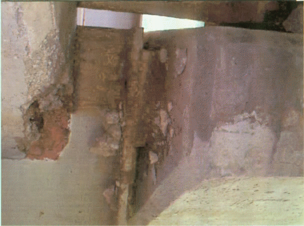
BT-3, SP-4; BUILDUP HAS H/L CRK UNDER BM-4 AND DIAPH IS SPALLED LT OF BM-4
