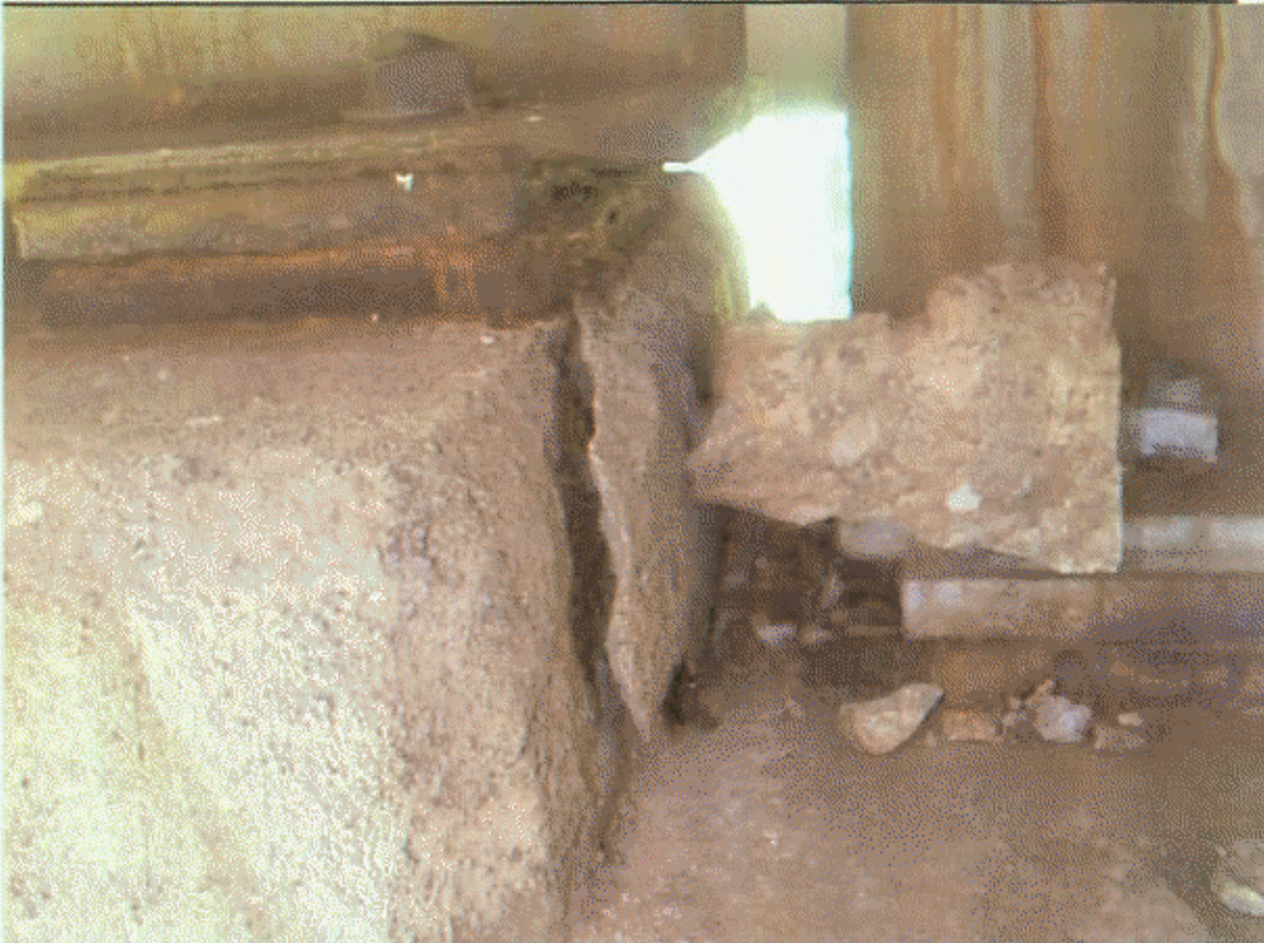
BT-2, SP-2; BUILDUP UNDER BM-4 HAS CRK TO 1/2" ON RT SIDE (SIMILAR CRK ON RT SIDE OF BM-5 UPTO 1/2", AT BTS 2 & 3)
