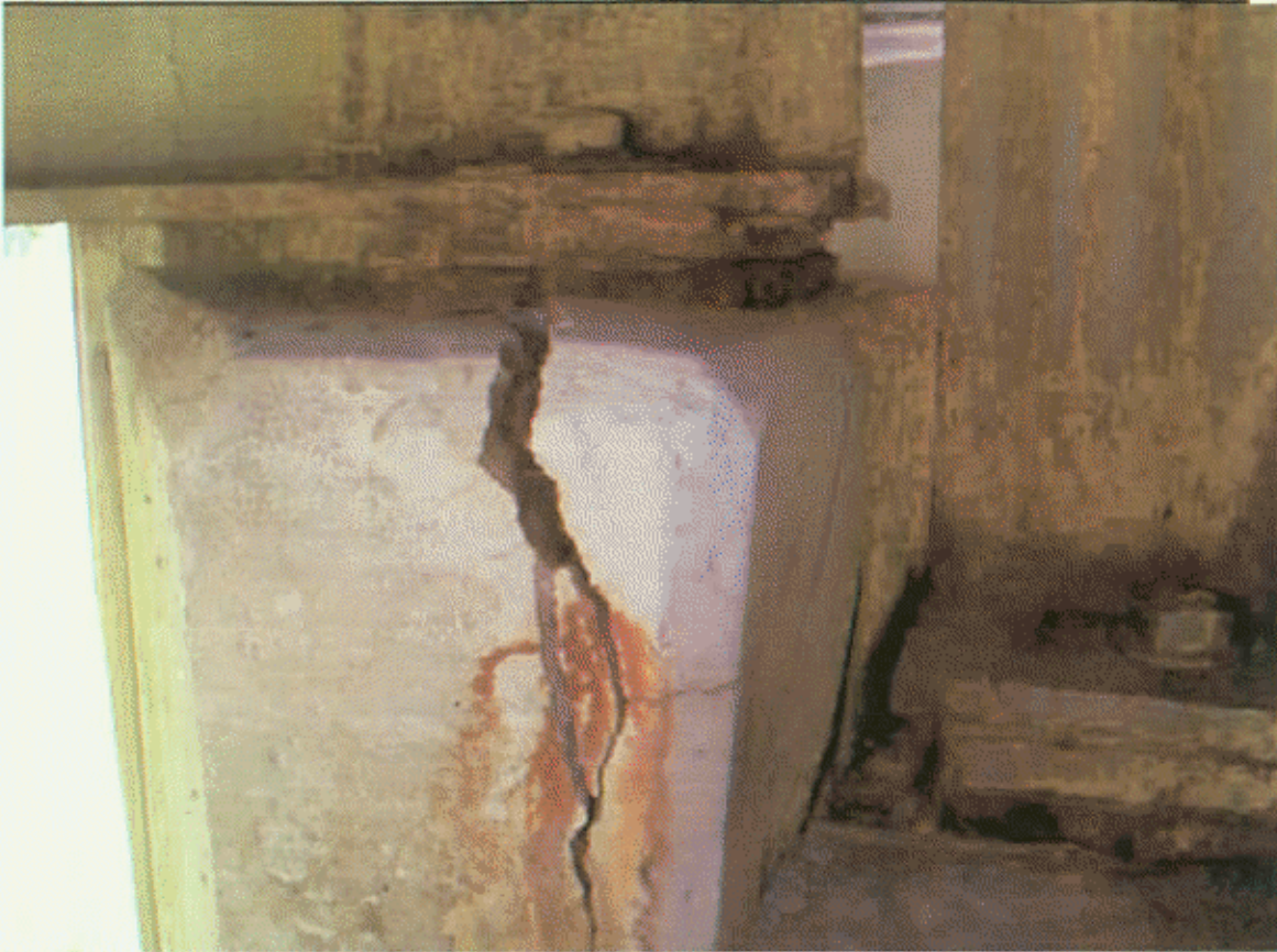
BT-3, SP-4; BUILDUP UNDER BM-2 HAS HORIZ CRK UPTO 3/4" ON LT SIDE AND BEARING HEAVILY RUSTED
