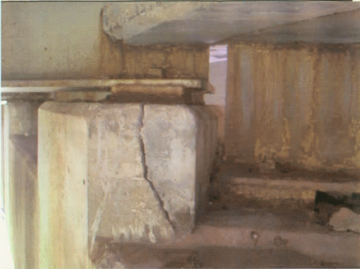
BT-3, SP-4; BUILDUP UNDER BM-3 HAS HORIZ CRK TO 1/2" WIDE ON LT SIDE
