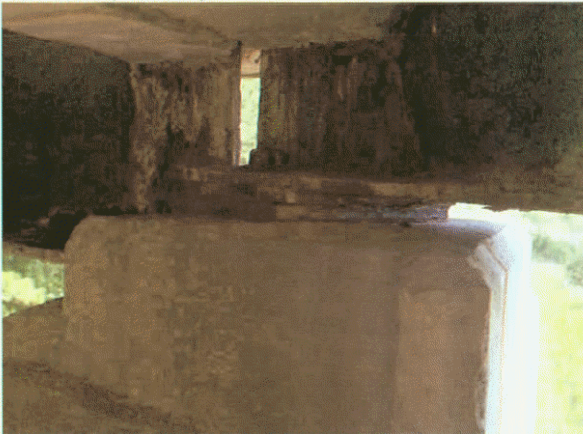
BT-2, BM-5 AND BEARINGS ARE HEAVILY RUSTED (OTHER EXTERIOR BEAMS SIMILAR)
