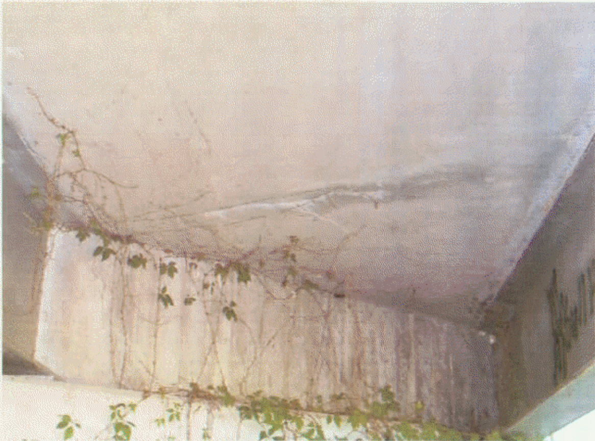
SP-5 AT END BT-2, BAY-4; DIAGONAL CRACKS W/EFFLO
