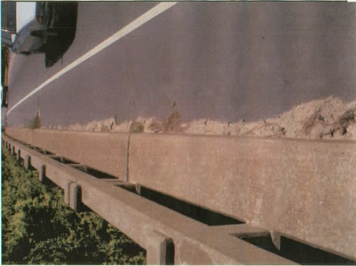
DEBRIS ALONG RT CURB (LT CURB)
