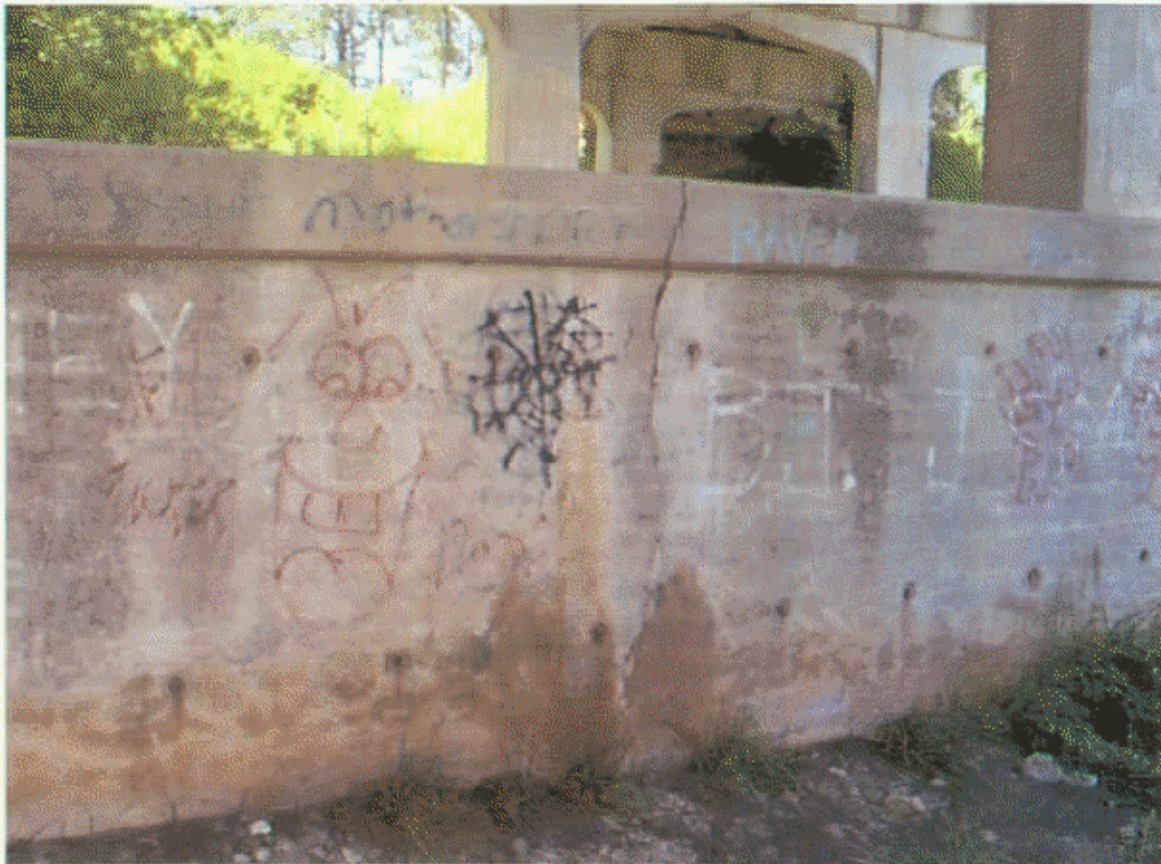
BT-2; PEDESTAL HAS VERTICAL CRKS TO 3/16" DOWN BOTH SIDES AND ACROSS TOP (BT-3 HAS SIMILAR CRACKING)
