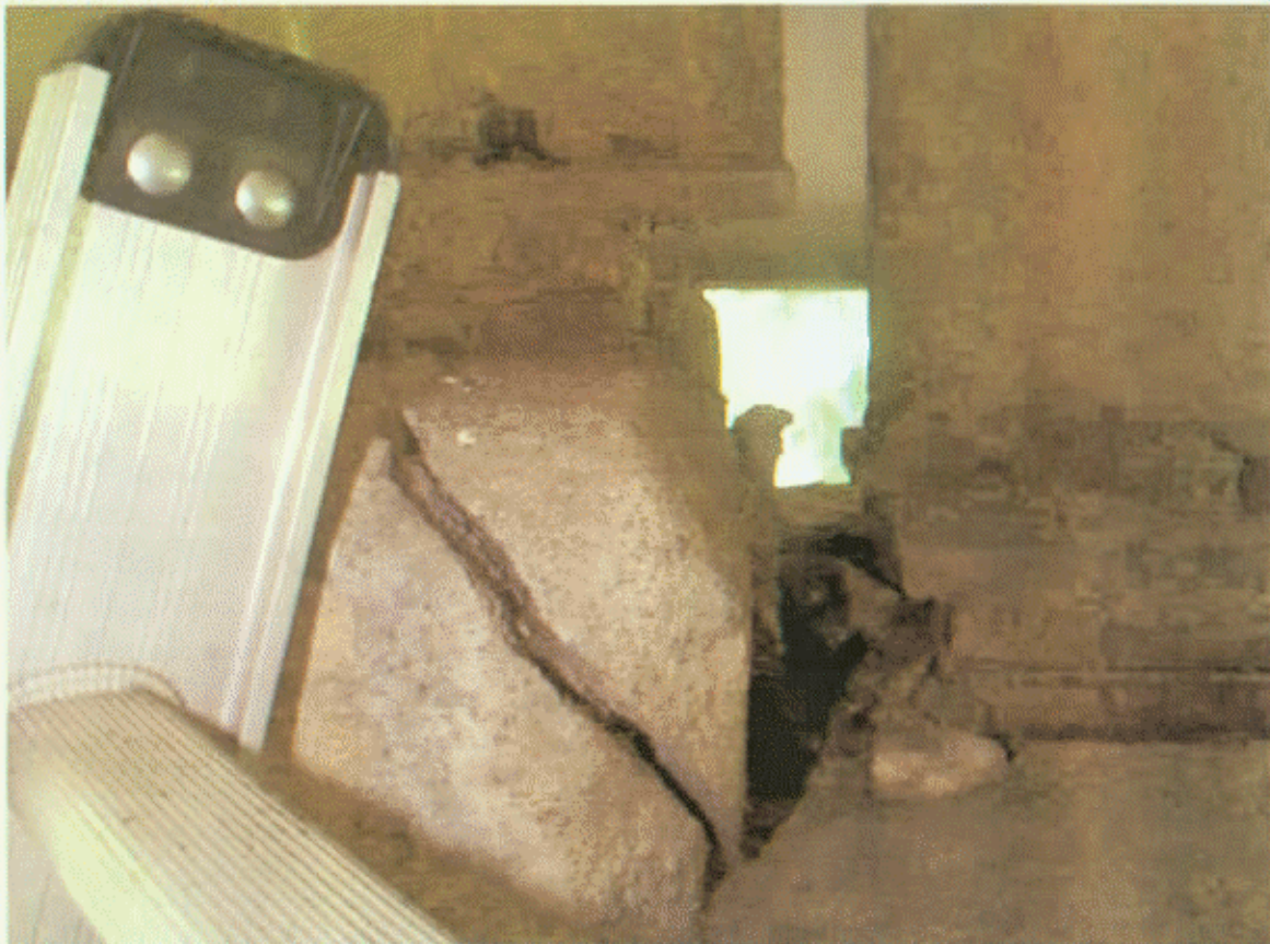
BT-2, SP-2; BUILDUP UNDER BM-2 IS CRKD TO 7/16" AND BEARING SLOTS FILLED W/RUST
