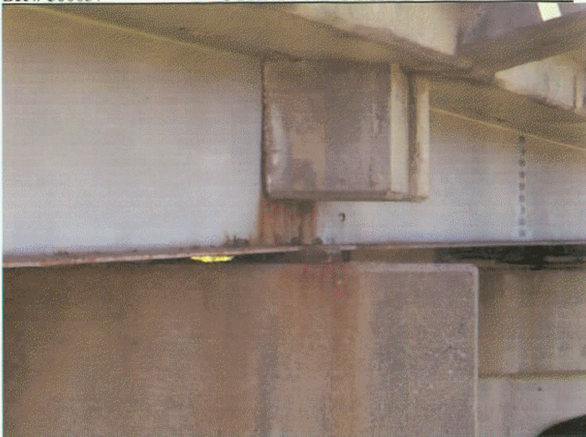
BT-1, RT EXTERIOR BEARINGS RUSTINGS (ALL EXTERIOR BEARINGS SIMILAR, ALSO RANDOM INTERIOR BEARINGS)
