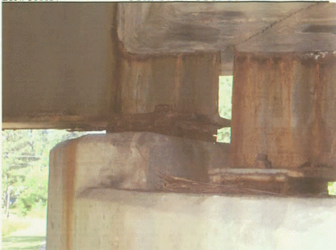
BT-2, SP-2; BM-1 BUILDUP IS CRKD TO 1/8" IN TWO PLACES
