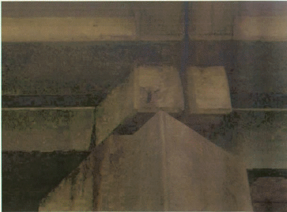
BT-3, SP-4; I.T EXTERIOR DIAPH SPALLED
