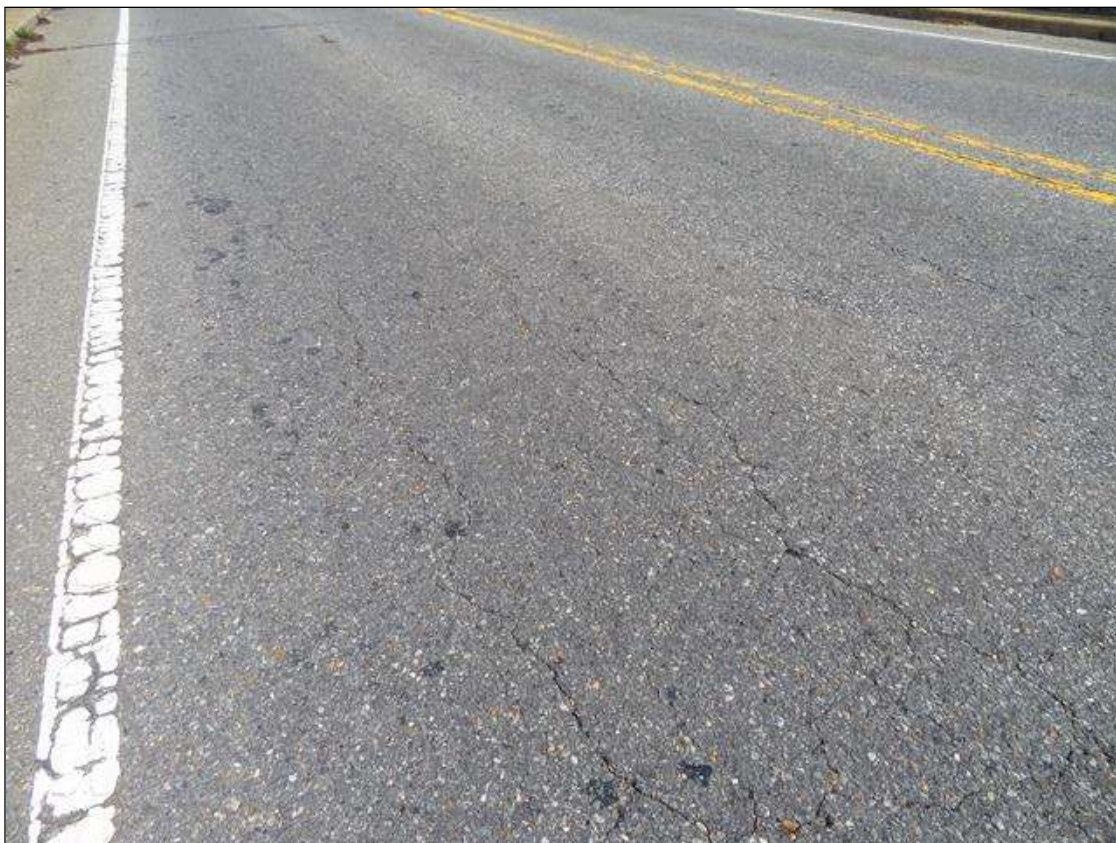
LONGITUDINAL CRACKING IN SPAN 2 WEARING SURFACE - OTHER SPANS SIMILAR
