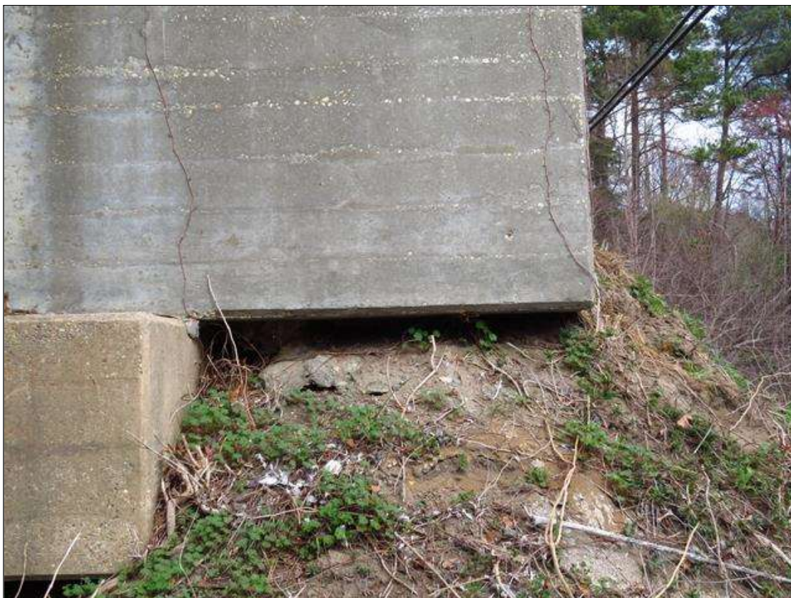
RIGHT END OF ABUTMENT 2 UNDERMINED 4' LONG X 10" HIGH X 12" DEEP
