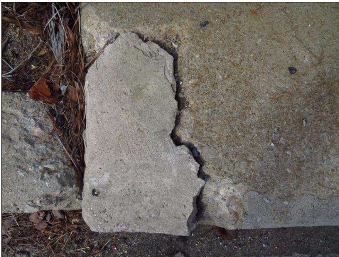
LEFT CURB AT END BENT 1 CRACKED AND SPALLED
