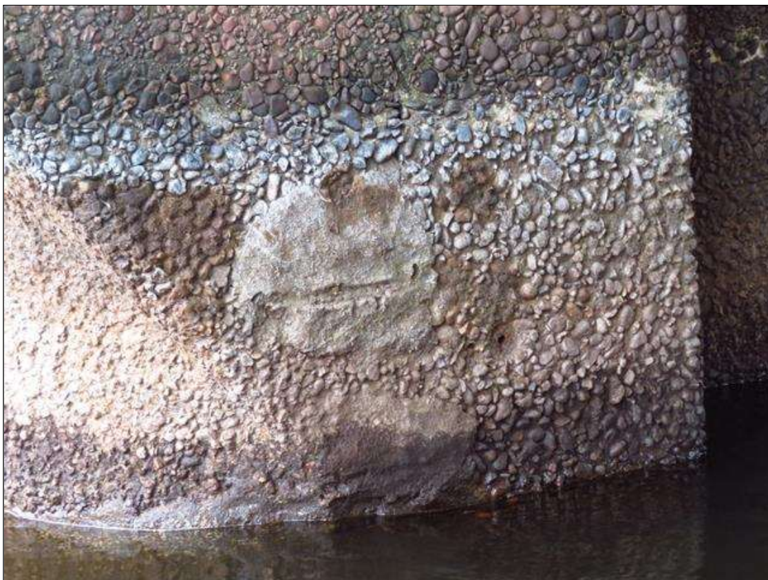
REPAIR PATCH IN SPAN 1 SIDE OF COLUMN 1 AT BENT 1 - COLUMN 2 SIMILAR
