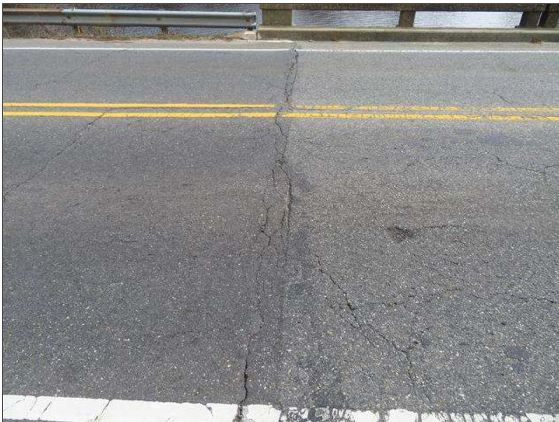
CRACKING IN WEARING SURFACE OVER END BENT 2
