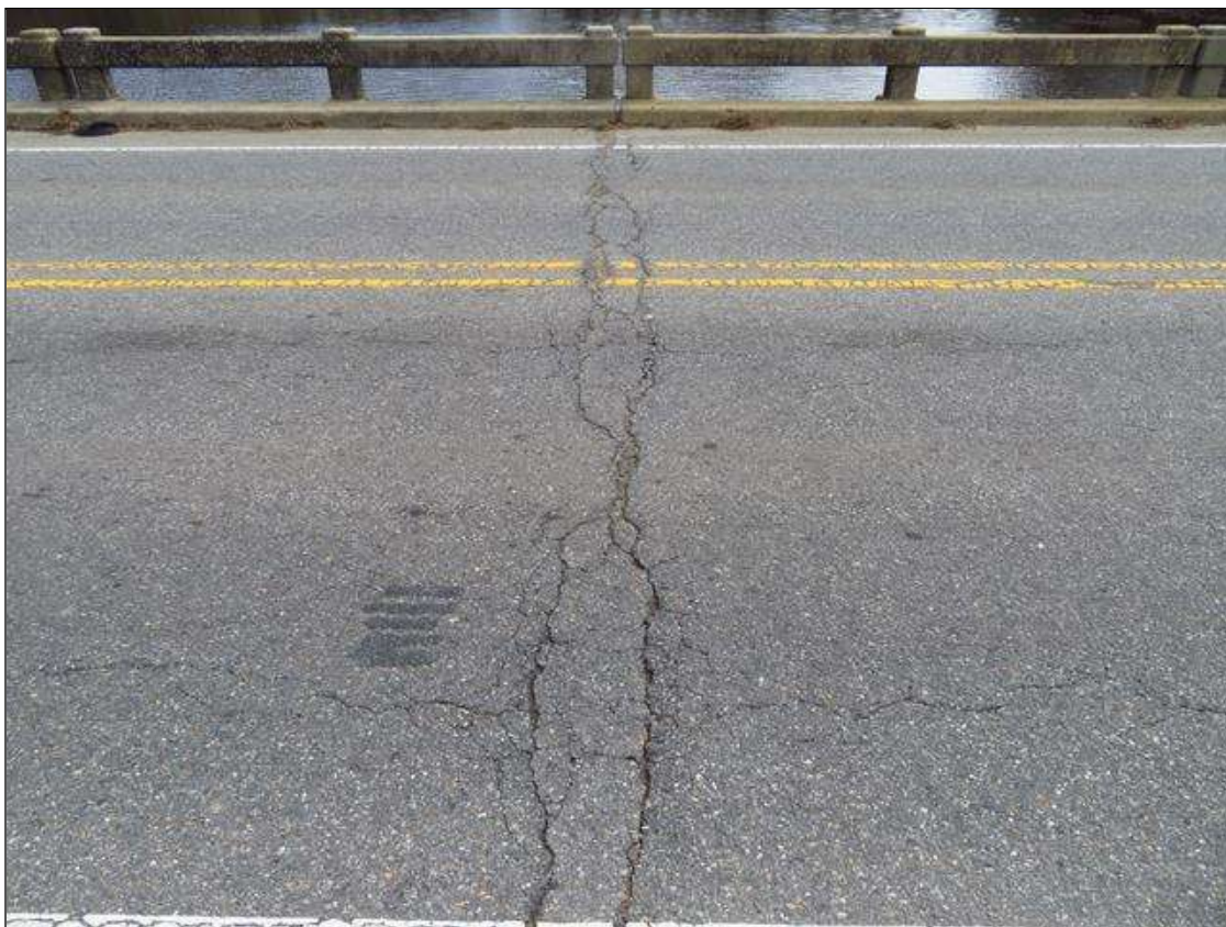
CRACKING IN WEARING SURFACE OVER BENT 3
