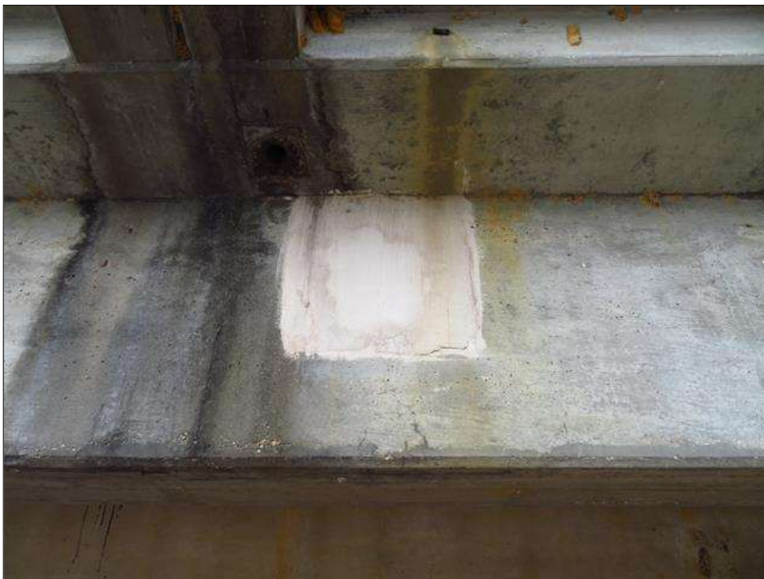
REPAIR PATCH IN THE RIGHT SIDE WEB OF GIRDER 5 IN SPAN 4 AT 2/3 POINT FROM BENT 3
