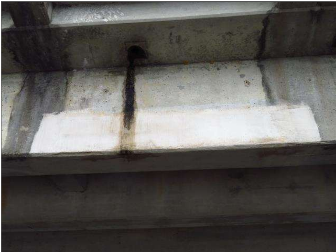
REPAIR PATCH IN THE RIGHT SIDE OF GIRDER 5 IN SPAN 2 AT MID-SPAN
