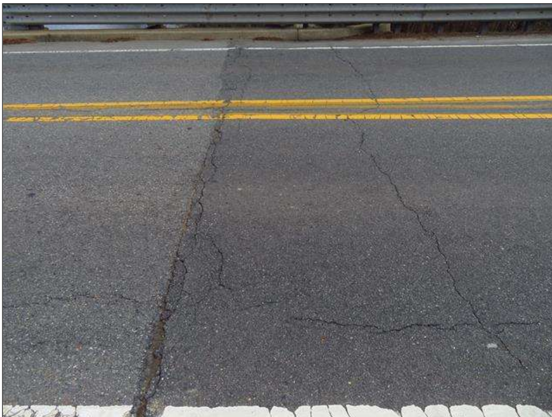
CRACKING IN WEARING SURFACE OVER END BENT 1
