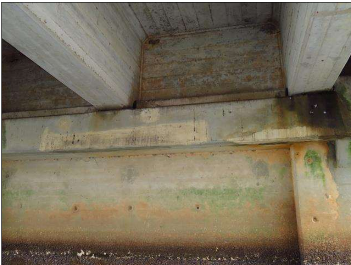
REPAIR PATCHING IN FACE OF CAP AT BENT 1 SPAN 1 SIDE UNDER GIRDERS 3 AND 4
