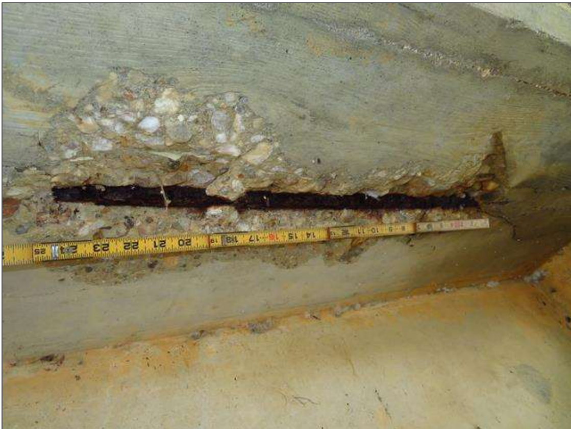
26" LONG X 7" WIDE X 2" DEEP SPALL WITH SECTION LOSS TO EXPOSED BAR IN BOTTOM OF CAP AT BENT 3 SPAN 3 SIDE UNDER BAY 4 (ESTIMATED 1" DIAMETER BAR REMAINING) PHOTO 1 OF 2
