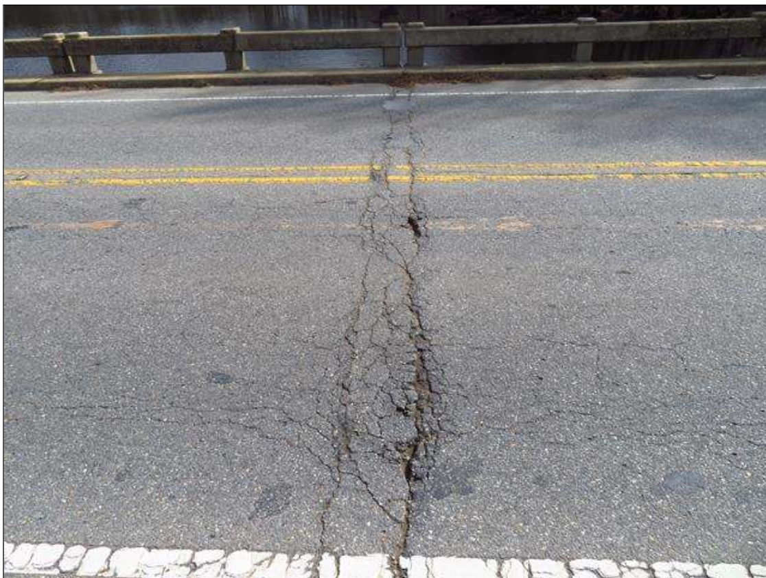
CRACKING IN WEARING SURFACE OVER BENT 1
