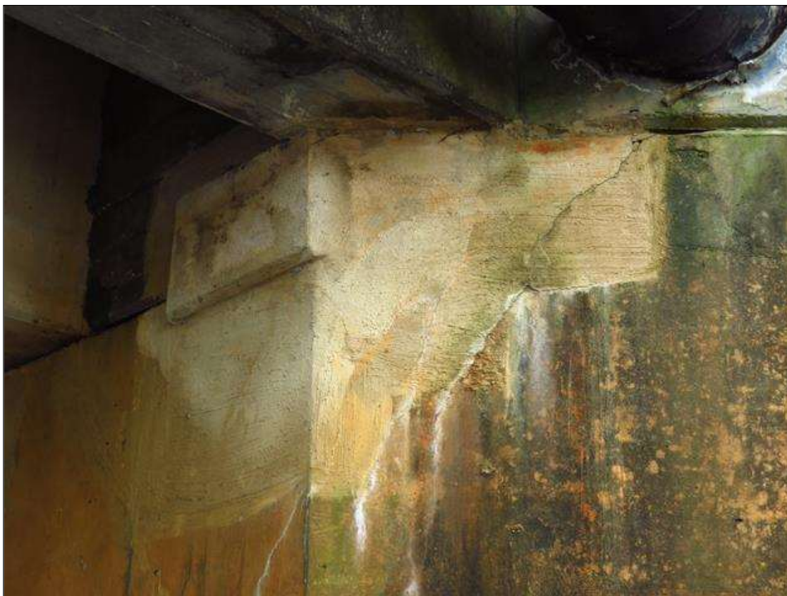
HAIRLINE TO 1/32" CRACK WITH SURFACE WHITE EFFLORESCENCE IN REPAIR PATCH IN ABUTMENT 1 AND IN CAP UNDER GIRDER 1
