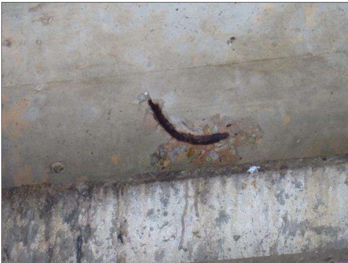
6" DIAMETER X 1" DEEP SPALL WITH EXPOSED REBAR IN SPAN 2 END DIAPHRAGM AT BENT 2 BAY 3
