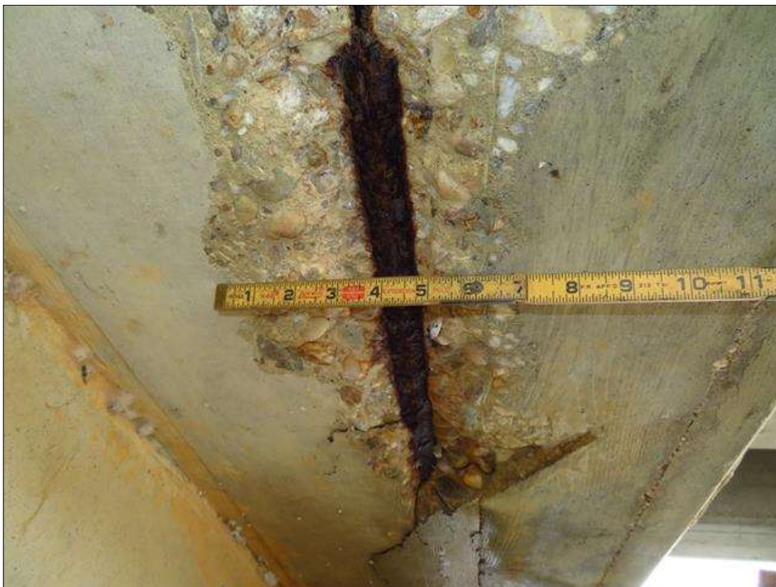
26" LONG X 7" WIDE X 2" DEEP SPALL WITH SECTION LOSS TO EXPOSED BAR IN BOTTOM OF CAP AT BENT 3 SPAN 3 SIDE UNDER BAY 4 (ESTIMATED 1" DIAMETER BAR REMAINING) PHOTO 2 OF 2
