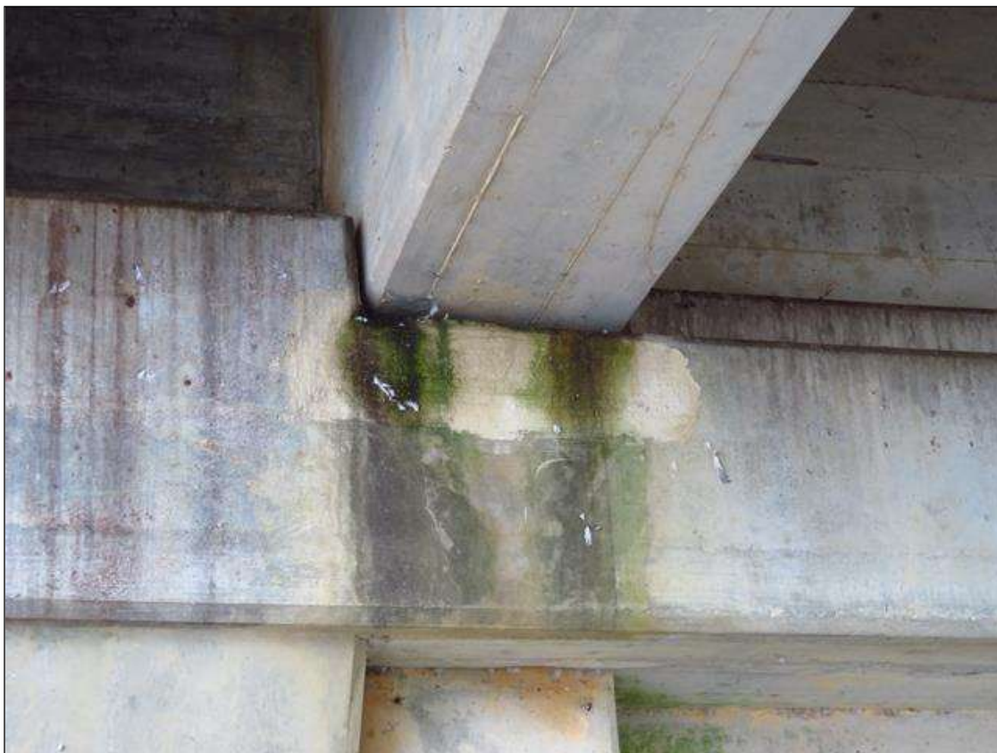
REPAIR PATCH IN FACE OF CAP AT BENT 3 SPAN 3 SIDE UNDER GIRDER 2
