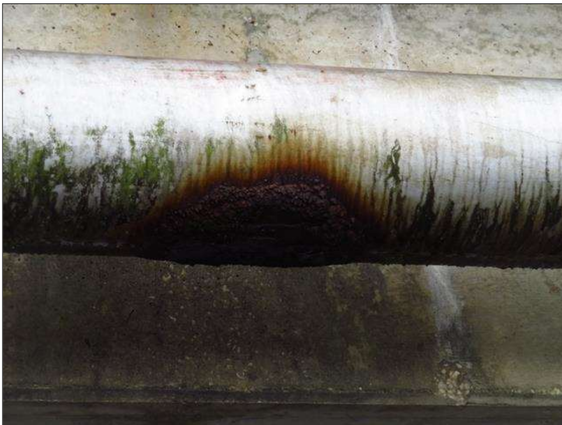
SPOTS OF CORROSION ALONG BOTTOM OF UTILITIES PIPE ALONG THE LEFT OVERHANG
