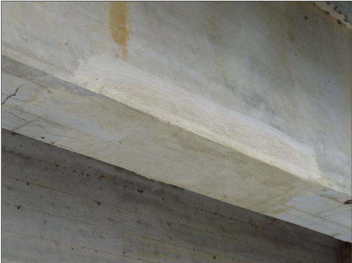
REPAIR PATCH IN THE BOTTOM OF GIRDER 4 IN SPAN 1 AT 2/3 POINT FROM ABUTMENT 1
