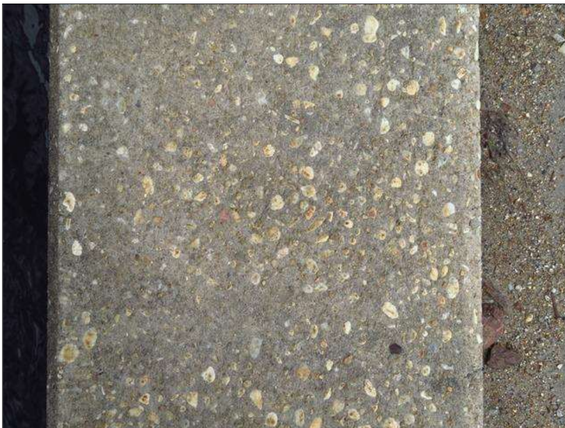
ABRASION WITH COARSE AGGREGATE EXPOSED ALONG DECK CURBS IN SPAN 2
