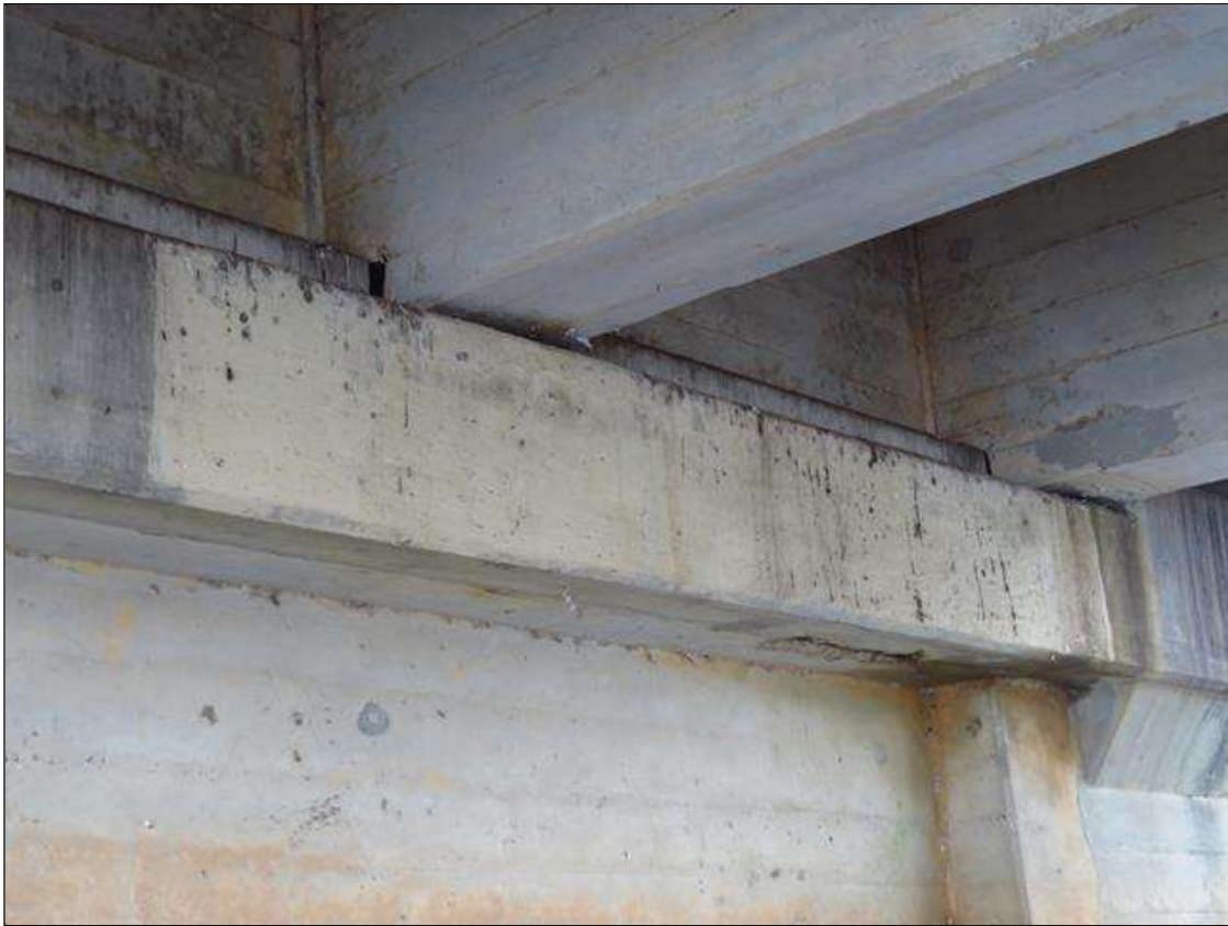
REPAIR PATCH IN FACE OF CAP AT BENT 3 SPAN 3 SIDE FROM GIRDER 3 TO GIRDER 4
