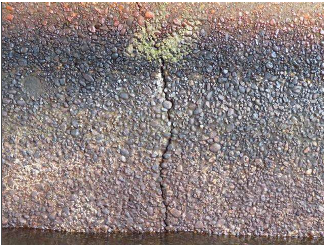
1/4" WIDE VERTICAL CRACK IN FACE OF ABUTMENT 1
