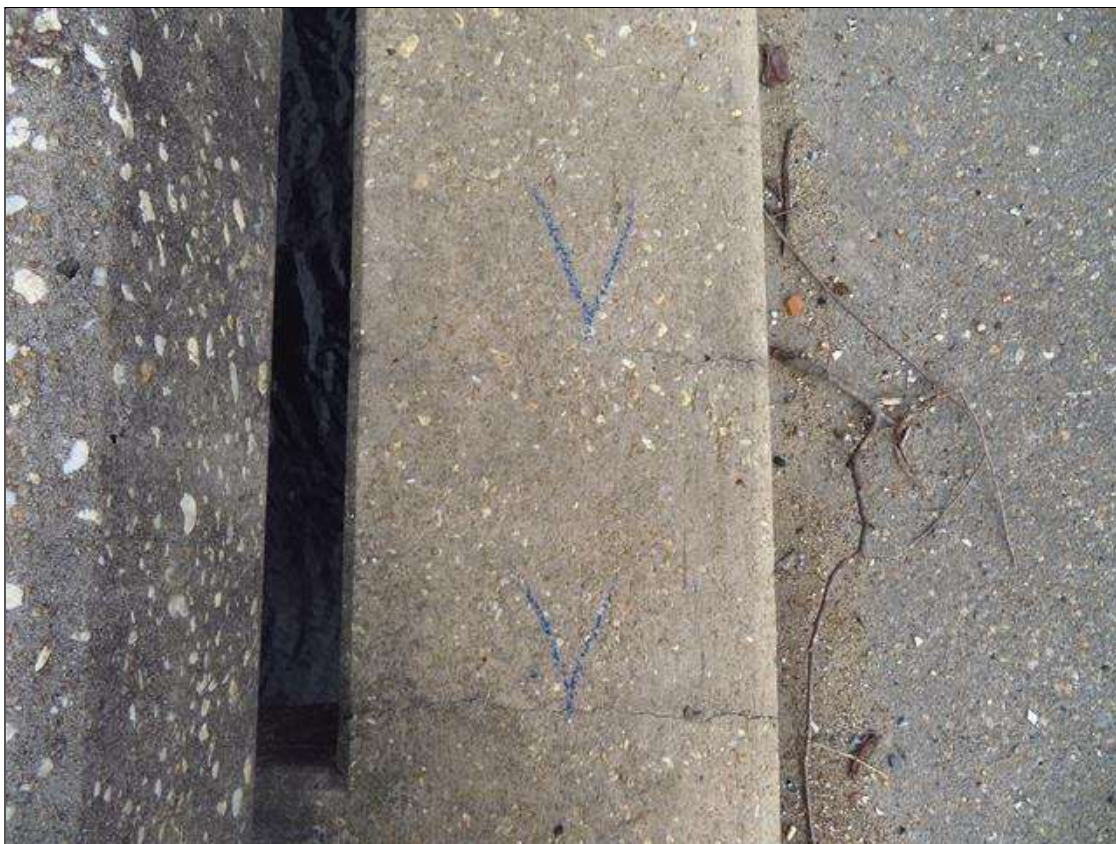
RANDOM TRANSVERSE CRACKS IN THE LEFT CURB OF SPAN 2
