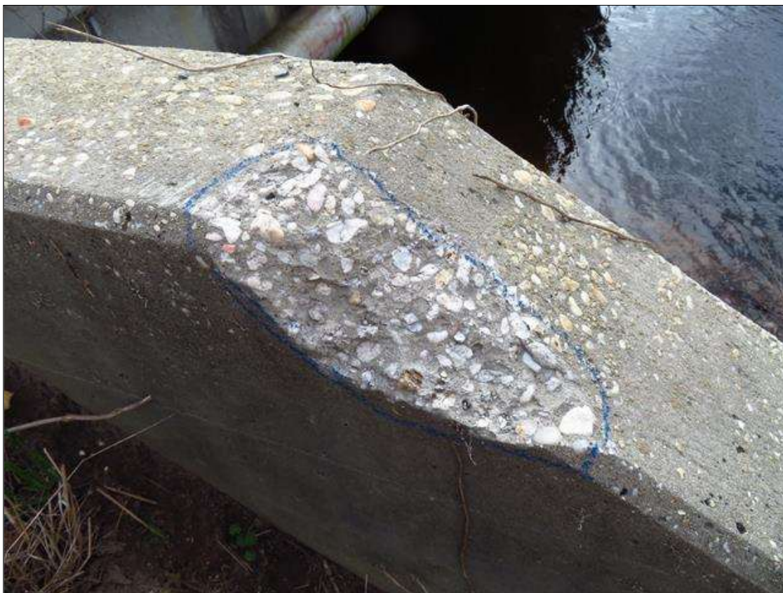
SPALL IN THE LEFT END OF ABUTMENT AT END BENT 2
