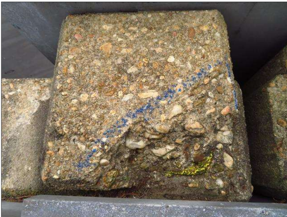
SPALL WITH EXPOSED REBAR IN THE RIGHT SIDE GUARDRAIL POST AT APPROACH GUARDRAIL CONNECTION IN SPAN 1
