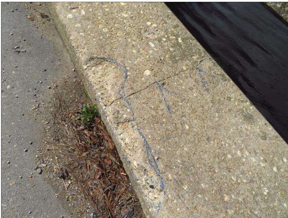
TRANSVERSE CRACK WITH SPALLING IN THE LEFT CURB OF SPAN 1
