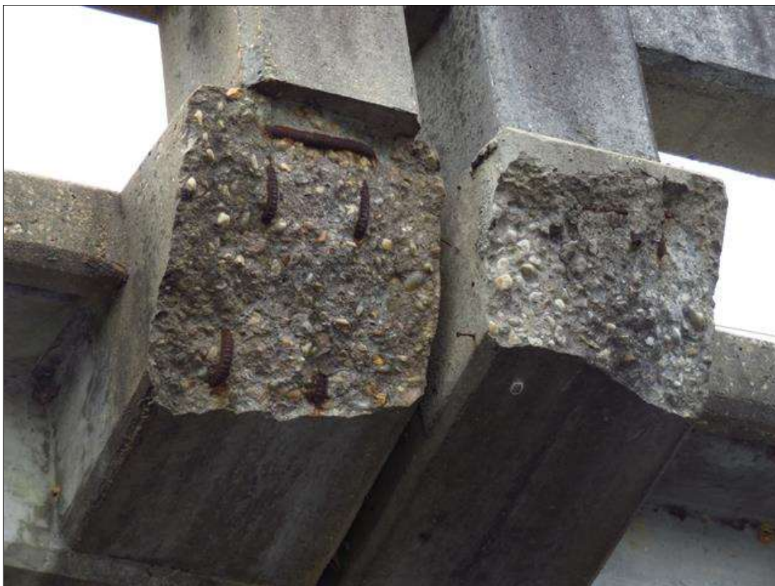
SPALLING WITH EXPOSED REBAR IN THE RIGHT SIDE DOG-EARS AT BENT 3
