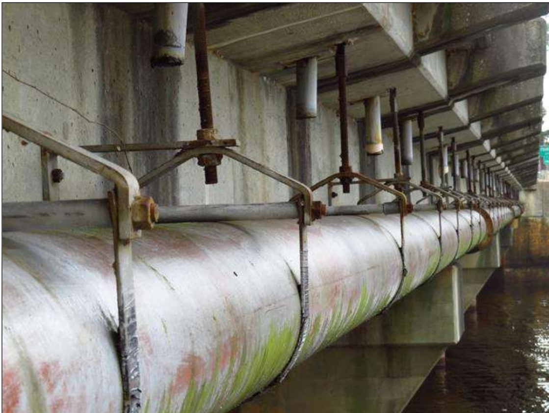
UTILITIES ALONG THE LEFT SIDE OVERHANG
