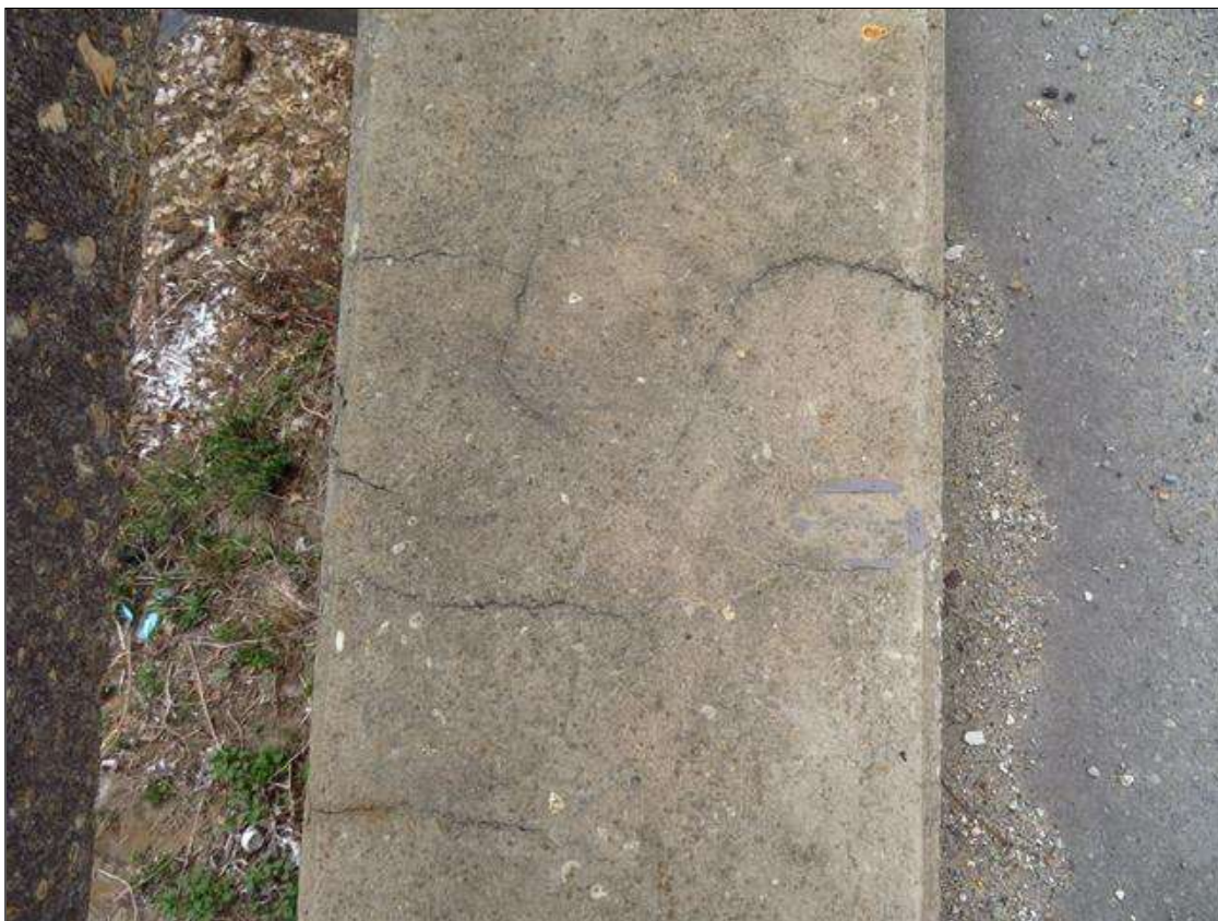
HAIRLINE CRACKING IN THE RIGHT CURB OF SPAN 4
