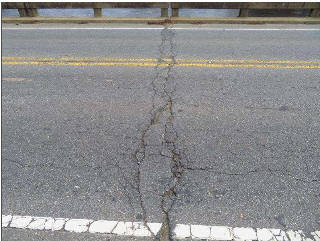
CRACKING IN WEARING SURFACE OVER BENT 2
