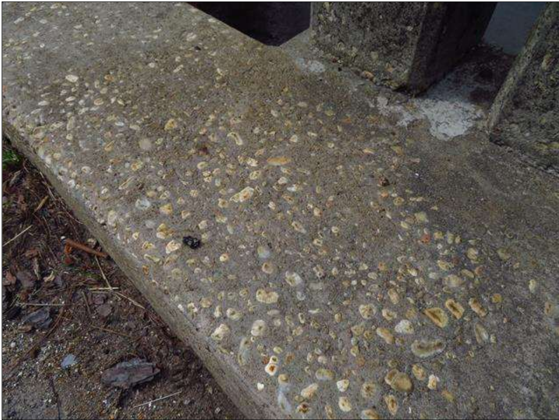
ABRASION WITH COARSE AGGREGATE EXPOSED ALONG DECK CURBS IN SPAN 1
