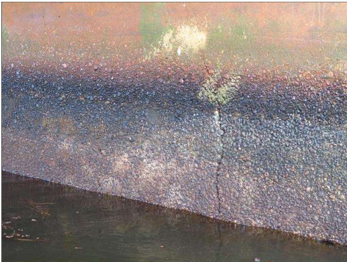
ABRASION WITH COARSE AGGREGATE EXPOSED FROM WATERLINE UP 3' AT ABUTMENT 1
