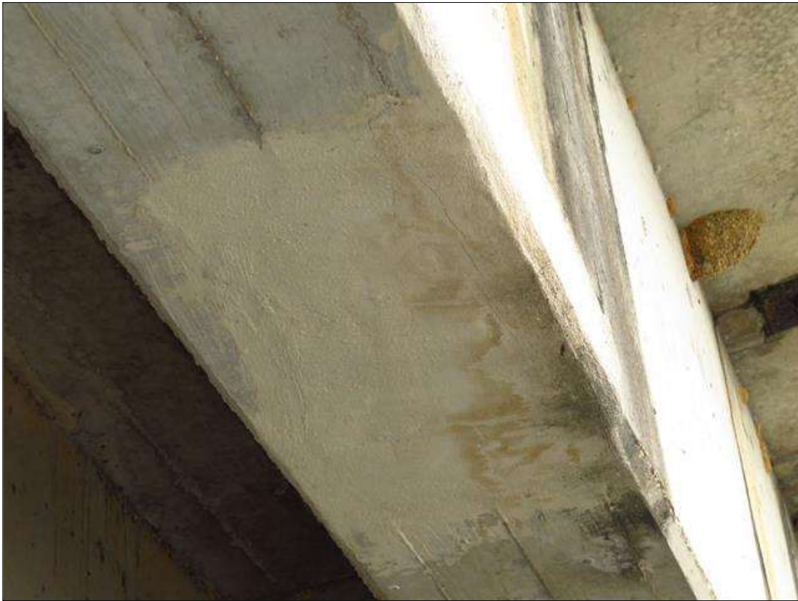
REPAIR PATCH IN THE BOTTOM OF GIRDER 5 IN SPAN 2 NEAR BENT 2
