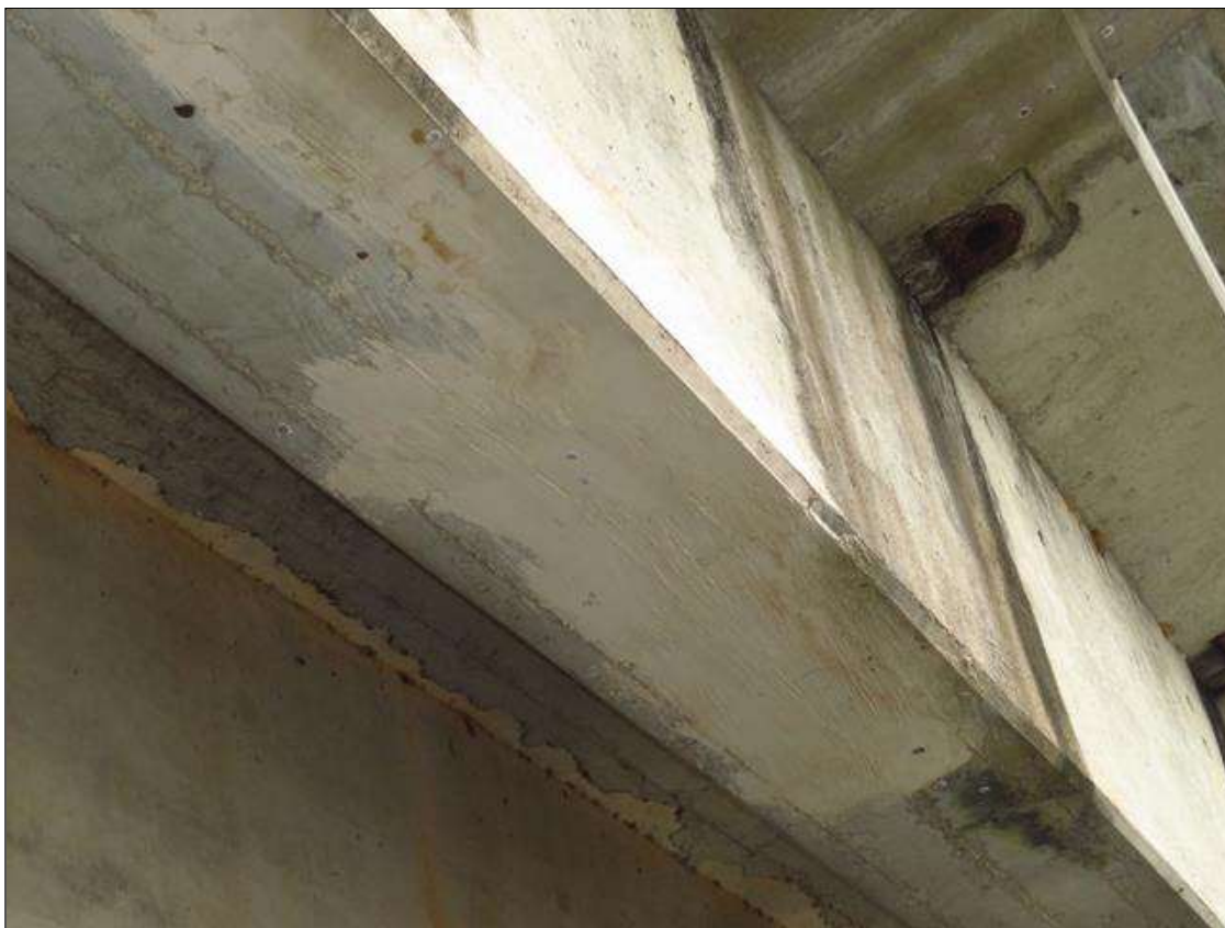
REPAIR PATCH IN THE BOTTOM OF GIRDER 5 IN SPAN 1 AT 2/3 POINT FROM ABUTMENT 1
