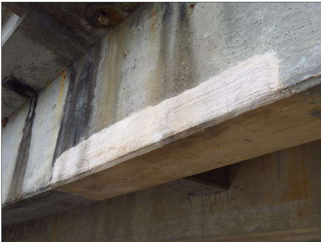
REPAIR PATCH IN THE RIGHT SIDE BOTTOM OF GIRDER 5 IN SPAN 4
