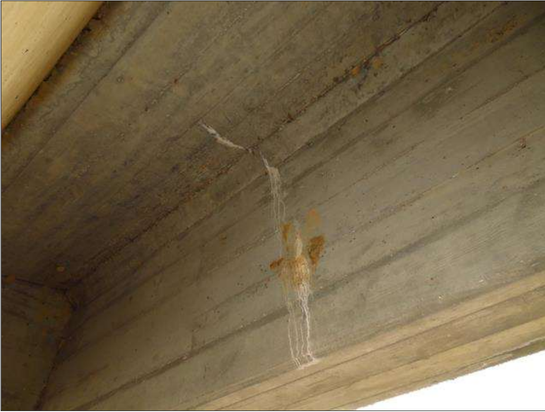
HAIRLINE CRACK WITH SURFACE WHITE EFFLORESCENCE IN BOTTOM OF DECK IN SPAN 4, BAY 1 EXTENDING DOWN THE RIGHT SIDE WEB OF GIRDER 1 NEAR MID-SPAN
