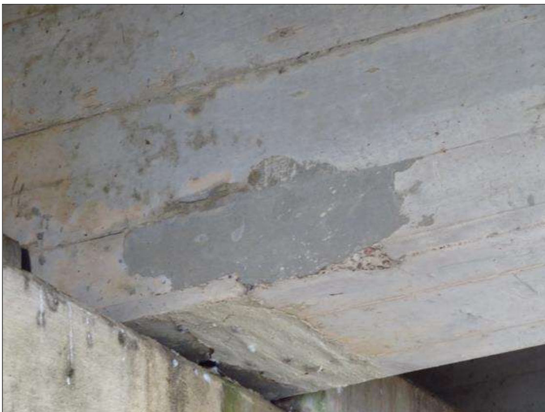
REPAIR PATCH IN THE LEFT SIDE OF GIRDER 4 IN SPAN 3 NEAR BENT 3
