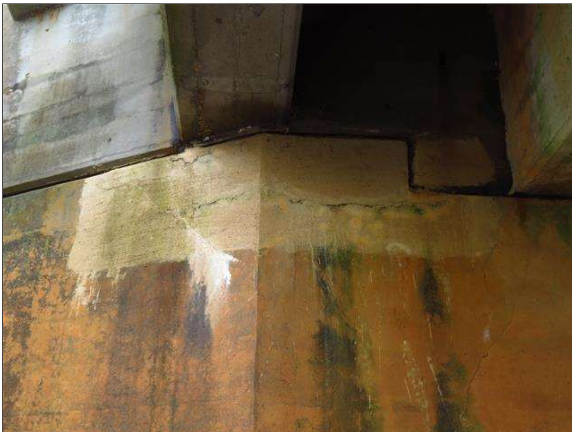
HAIRLINE CRACK WITH SURFACE WHITE EFFLORESCENCE IN REPAIR PATCH IN ABUTMENT 1 AND IN CAP UNDER GIRDER 5
