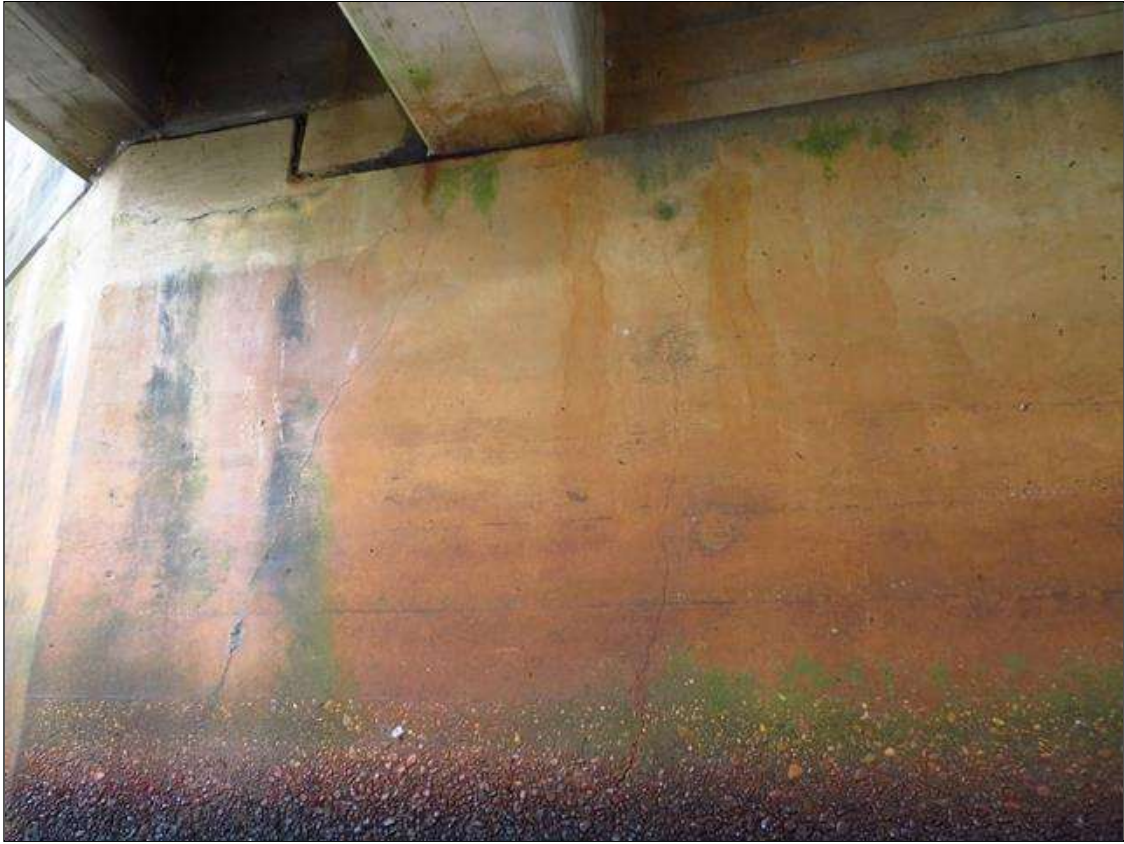
VERTICAL CRACKS IN FACE OF ABUTMENT 1 UNDER GIRDER 4
