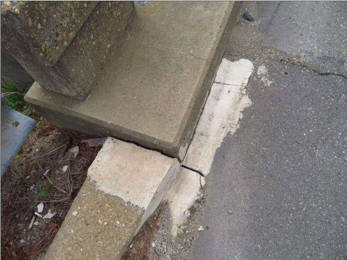
REPAIR PATCH IN THE RIGHT SHOULDER AND CURB AT END BENT 2
