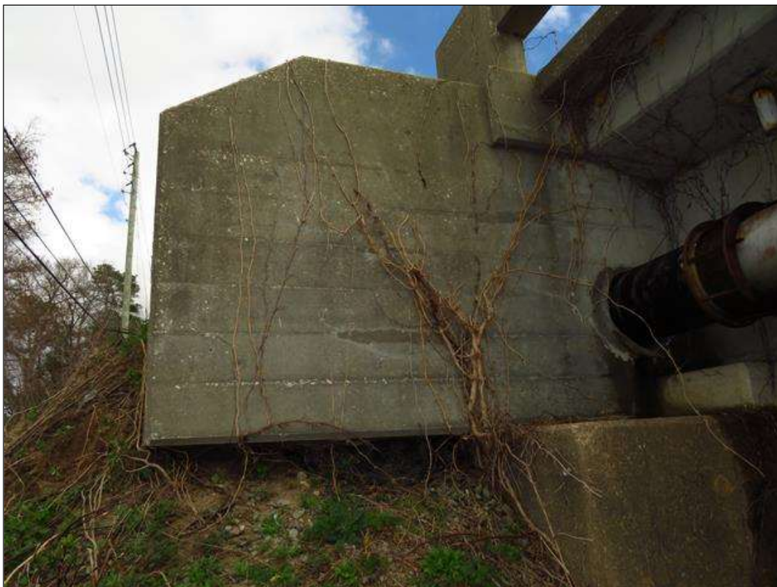
LEFT END OF ABUTMENT 2 UNDERMINED 4'L X 10" HIGH X 10" DEEP
