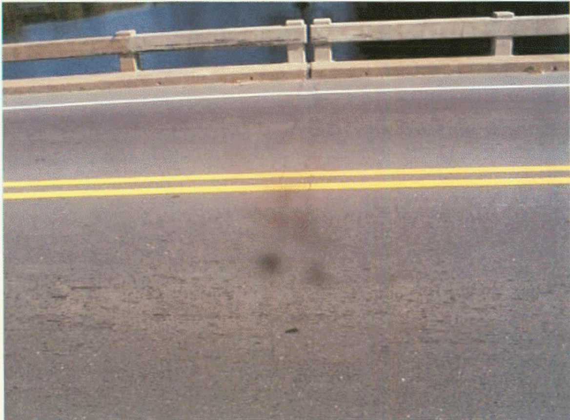
ASPHALT WEARING SURFACE AT BENT 1 JOINT
