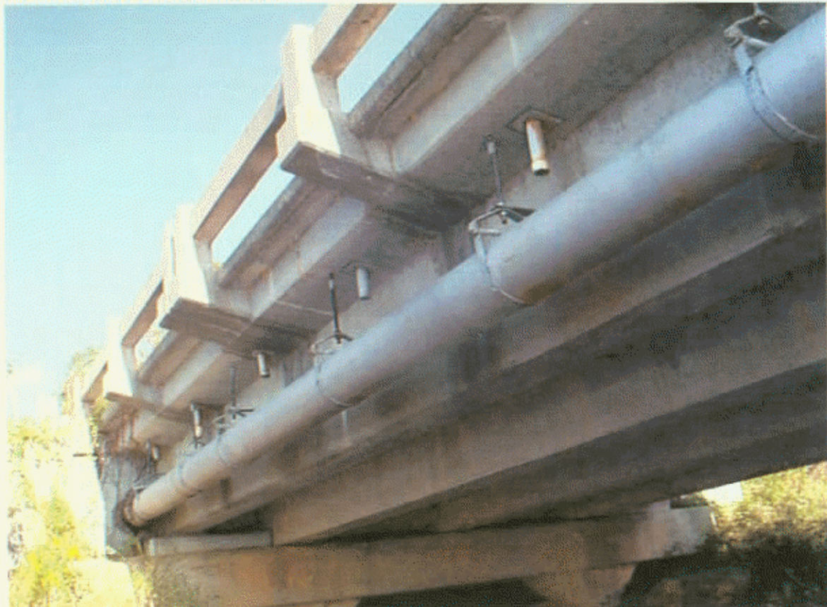
WEST SIDE UTILITY
