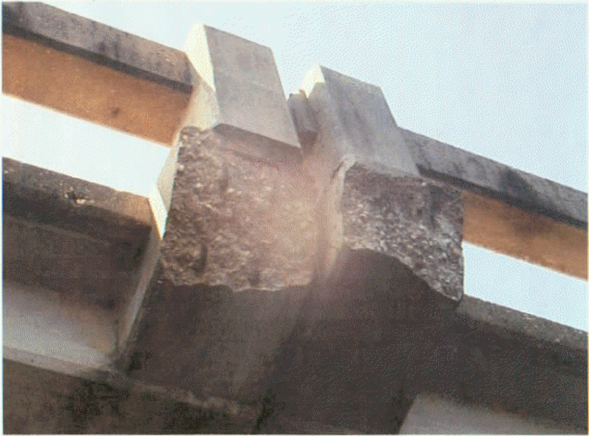
EAST RAIL POST @ BENT 3 SPALLED AT UNDERSIDE
