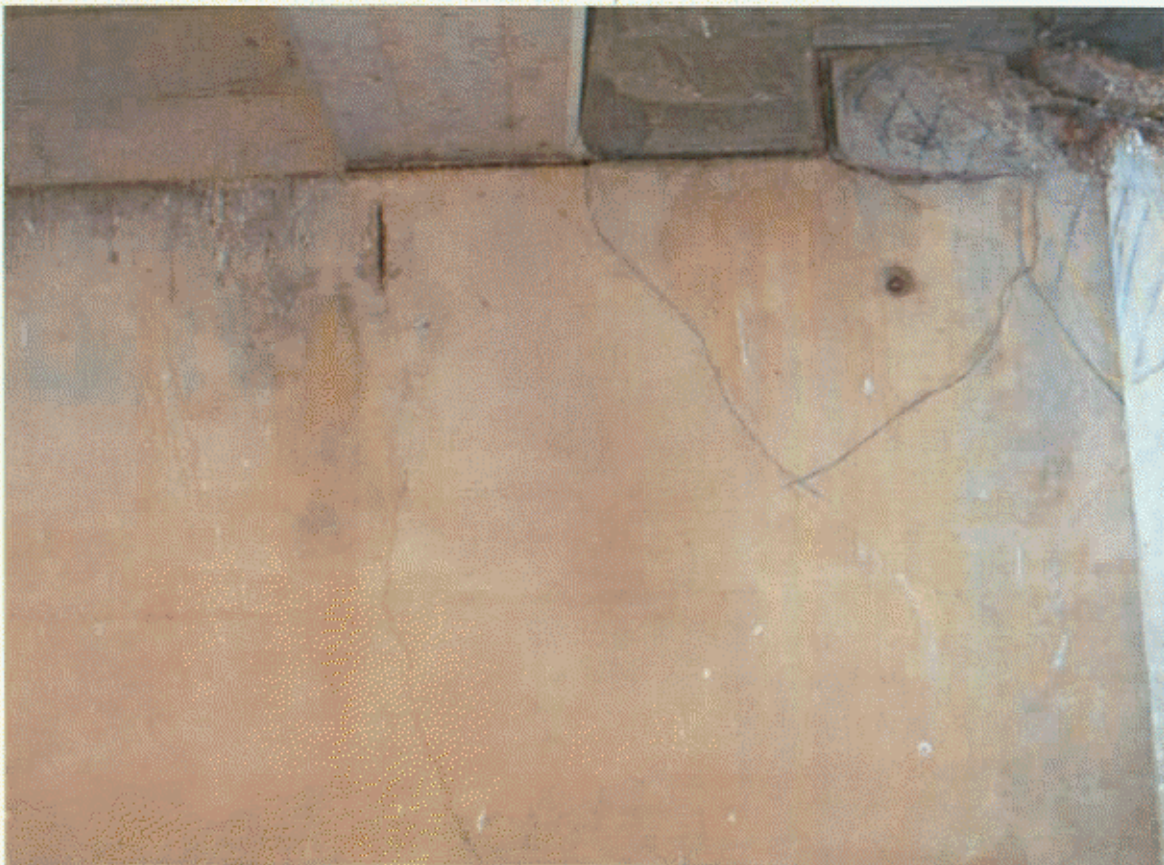
CRACKED & DELAM. AT GIRDER 2, ABUT. 1
