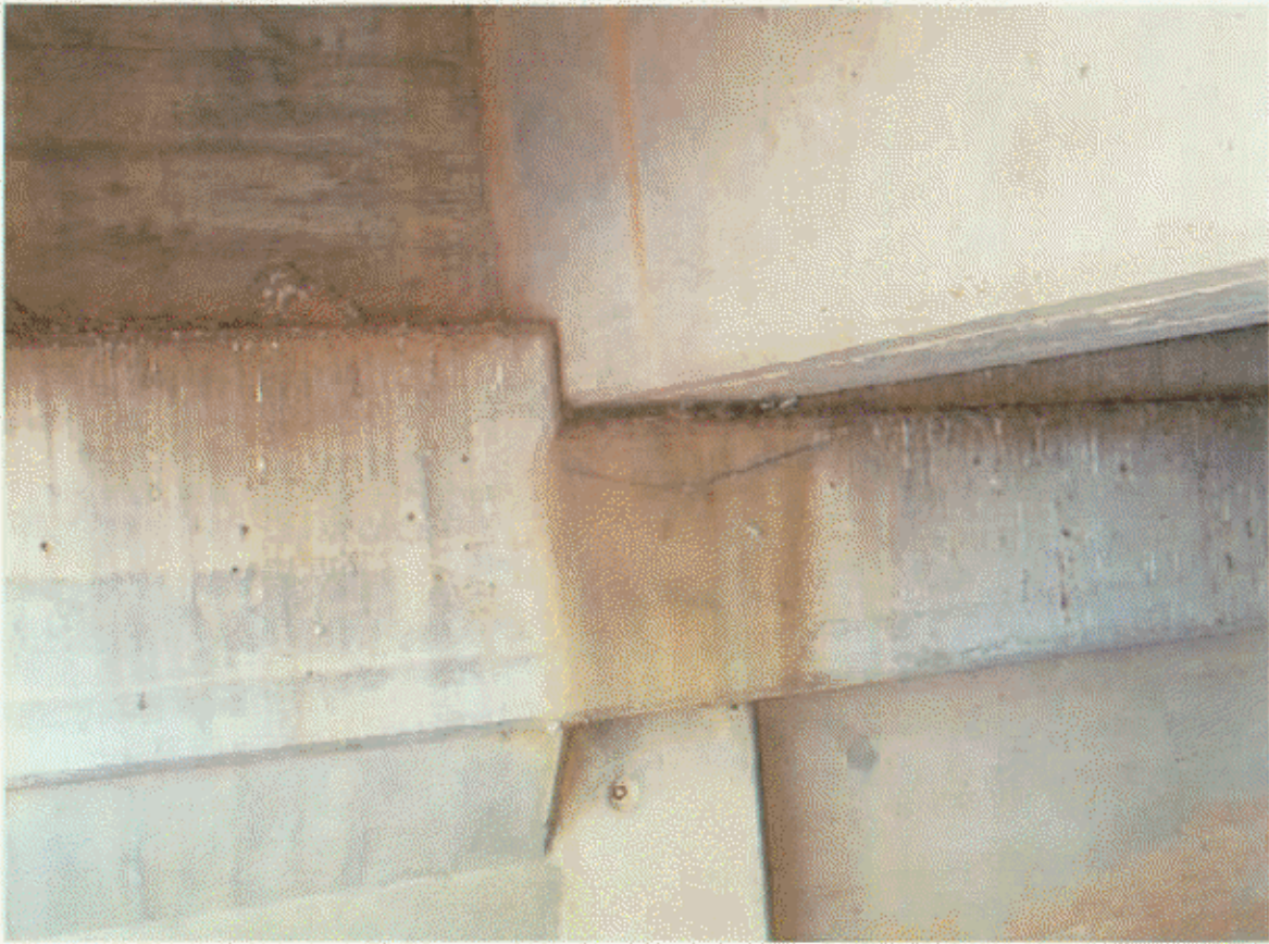
BENT 3 AT GIRDER 1, SPAN 3 CRACKED & DELAM.
