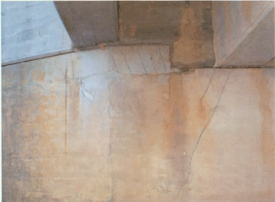
CRACKED & DELAM. AT GIRDER 5, ABUT. 1
