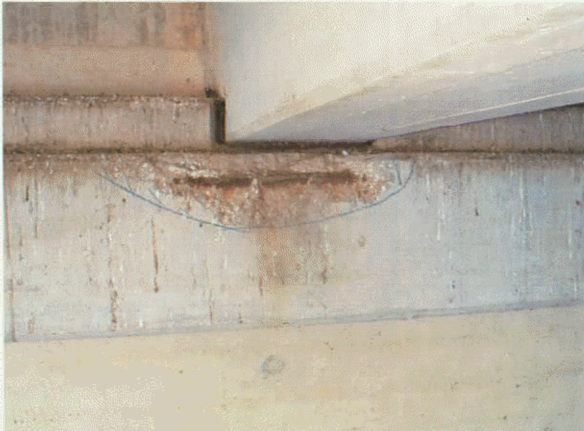
BENT 3 AT GIRDER 2, SPAN 3 SPALLED W/ EXPOSED REBAR
