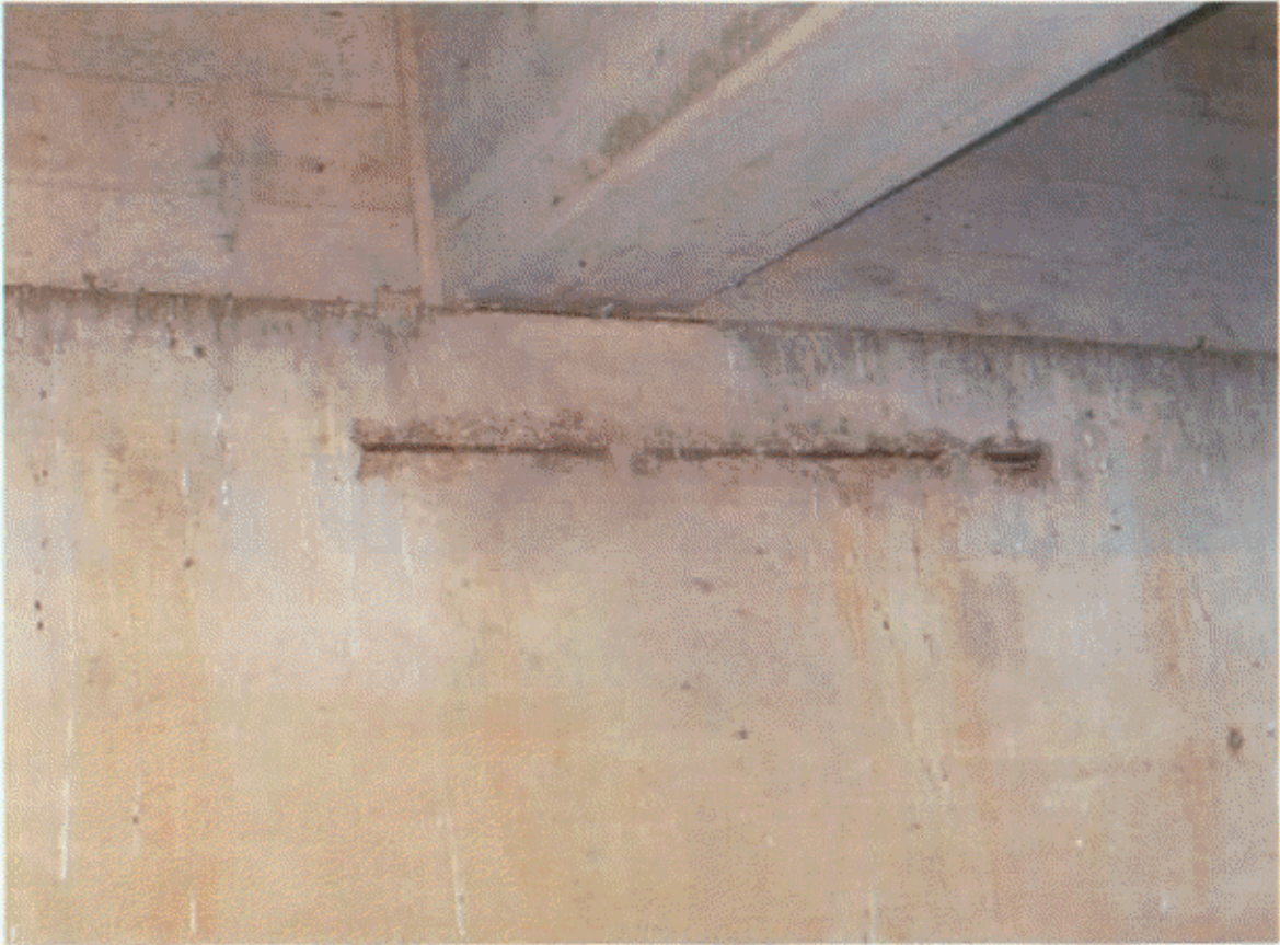
SPALLED W/ EXPOSED REBAR AT GIRDER 3, ABUT. 1
