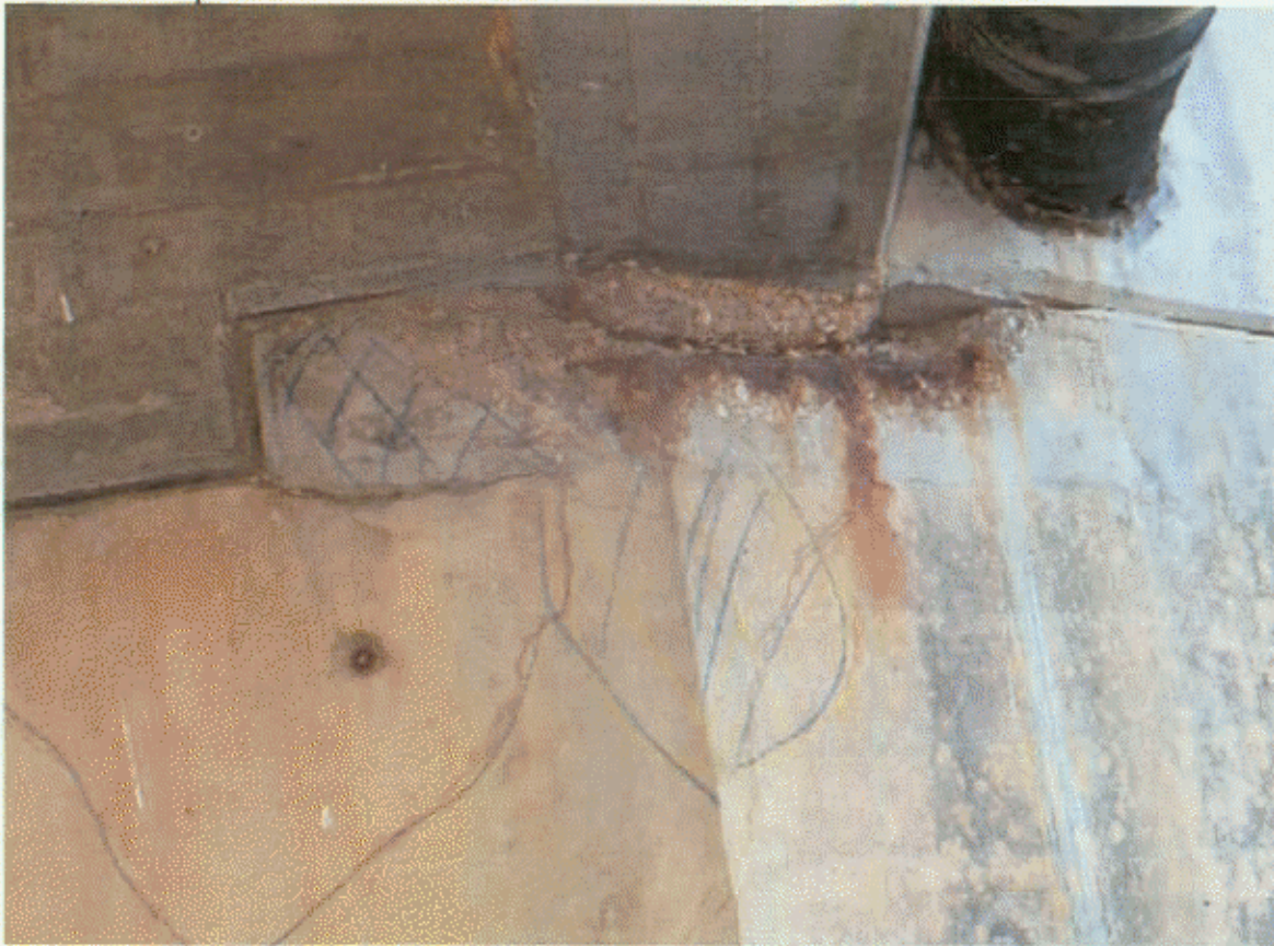
CRACKED & DELAM. AT GIRDER 1, ABUT. 1
