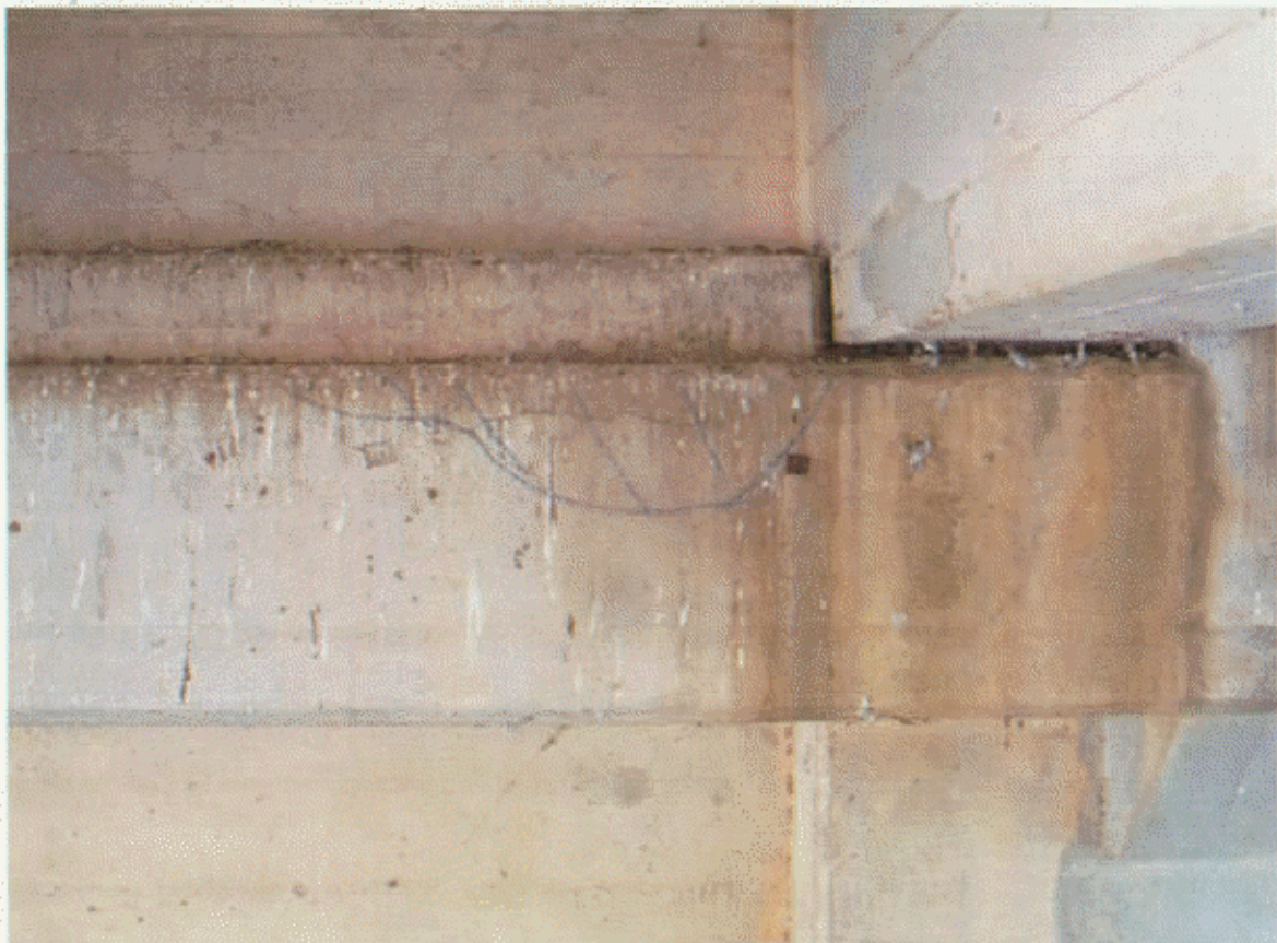
BENT 3 AT GIRDER 3, SPAN 3 CRACKED AND DELAM.
