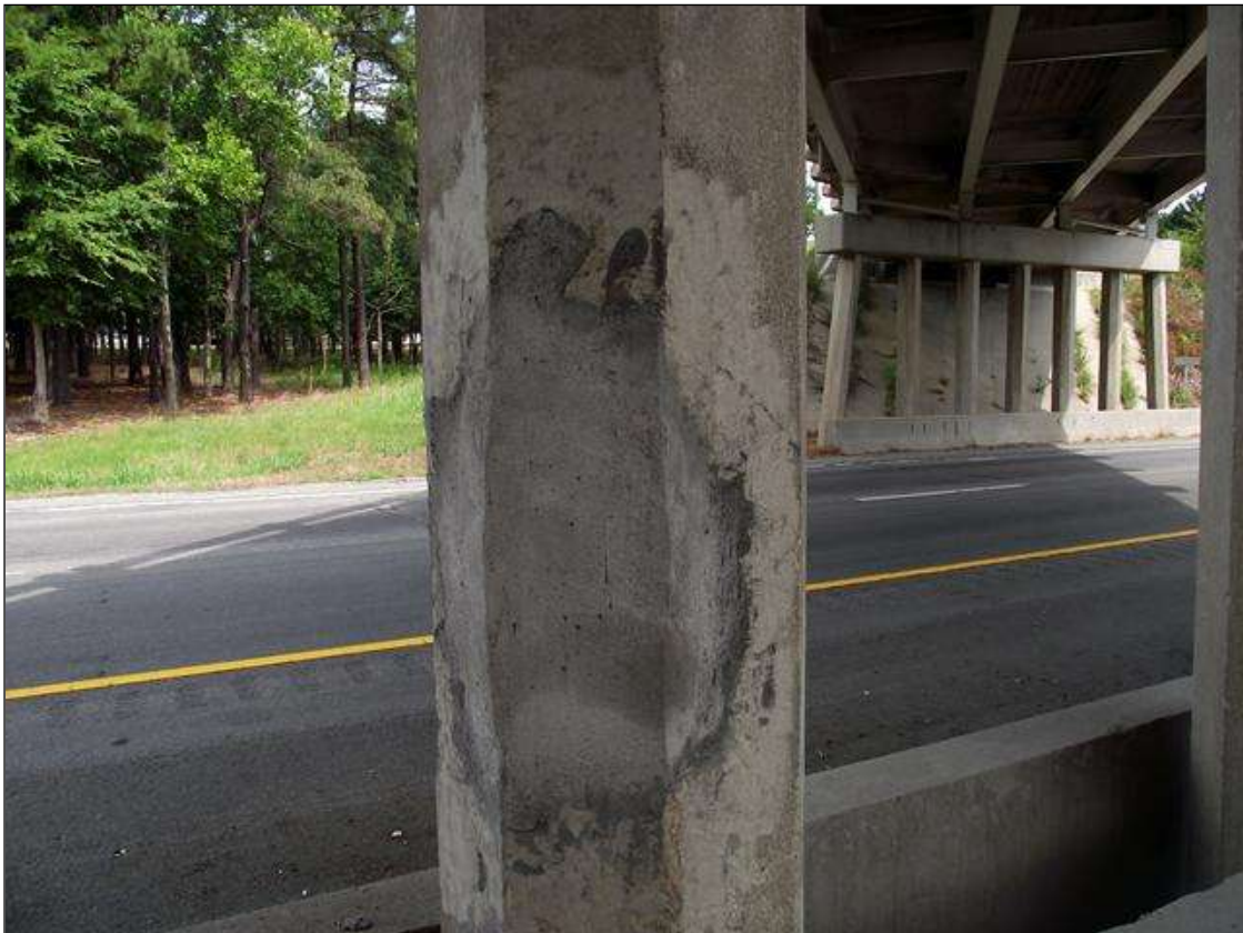
SPALL REPAIR IN FACES 1, 2 & 3 OF PILE NO.2 AT BENT 2
