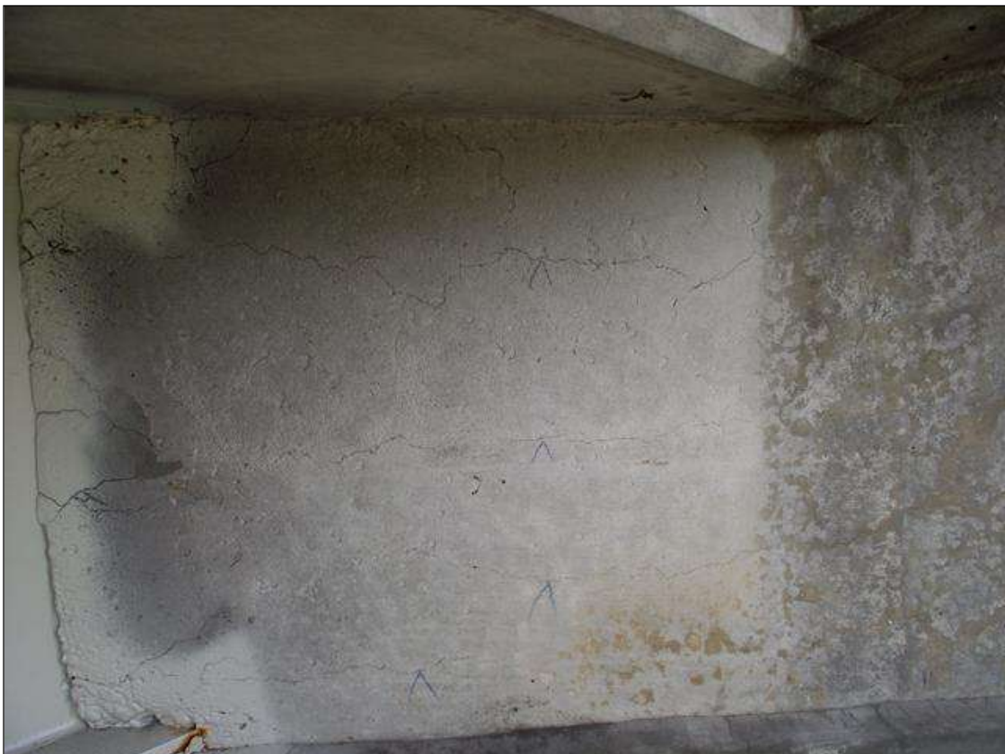
HORIZONTAL CRACKS IN LEFT BACKWALL EXTENSION AT END BENT 1
