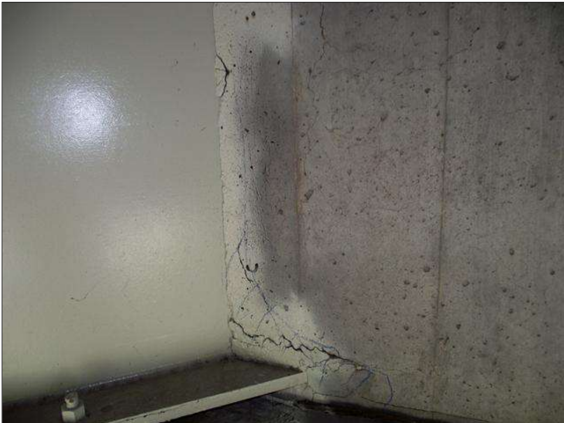
DELAMINATION IN ORIGINAL BACKWALL AT END BENT 1 LEFT OF BEAM 2
