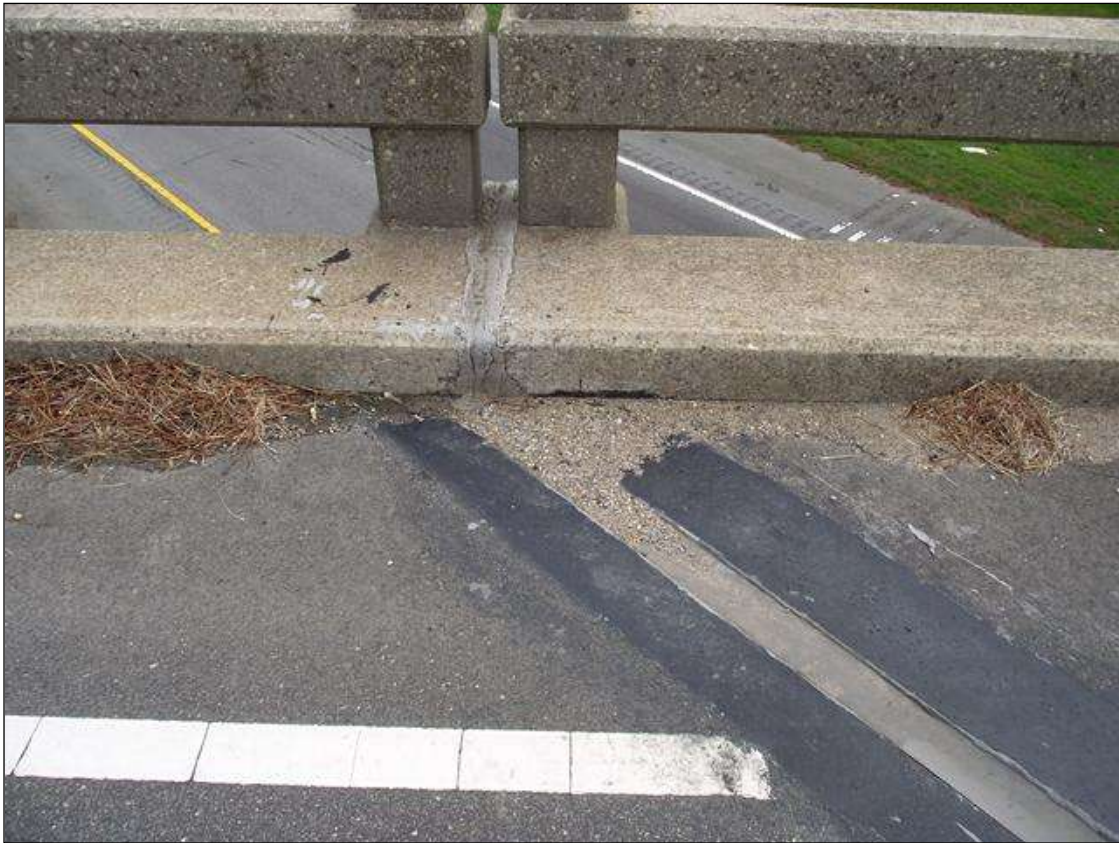
DIRT AND DEBRIS IN SHOULDERS AT EXPANSION JOINTS
