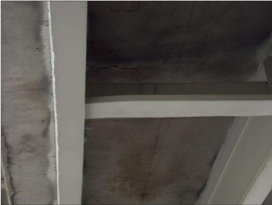
INTERIOR DIAPHRAGM IN SPAN 2 BAY 1 AT 1/3 POINT IS BENT FROM PREVIOUS IMPACT DAMAGE
