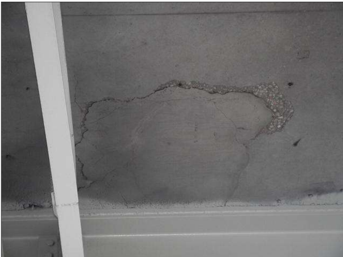
PATCH IN BOTTOM OF DECK OF SPAN 2 BAY 1 AT 1/3 POINT
