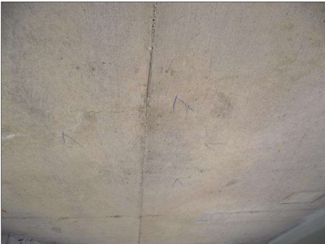
HAIRLINE TO 1/32 IN. MAP CRACKING IN BOTTOM OF DECK OF SPAN 1 BAY 1 - OTHER BAYS SIMILAR
