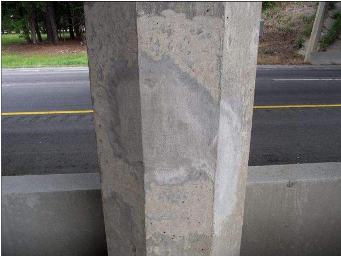
SPALL REPAIR IN FACES 1, 2 & 8 IN PILE NO.4 AT BENT 2
