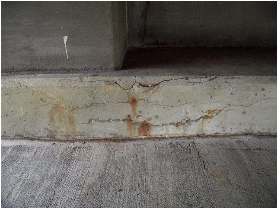
CRACKING AND DELAMINATION WITH RUST STAINS IN FACE OF CAP AT END BENT 2 BAY 1
