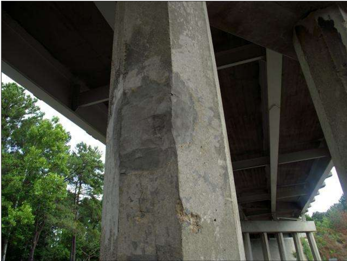
SPALL REPAIR IN FACES 1 & 2 OF PILE NO.4 AT BENT 2
