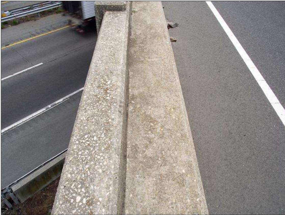
CURBLINES AND GUARDRAILS ARE WEATHERED WITH COARSE AGGREGATE EXPOSED
