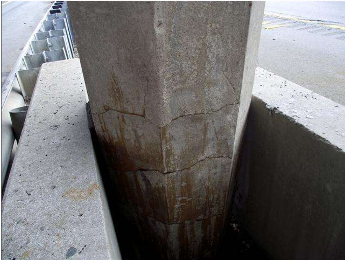
HORIZONTAL CRACKS IN FACES 1, 2, 3, 4 & 5 OF PILE NO.6 AT BENT 2
