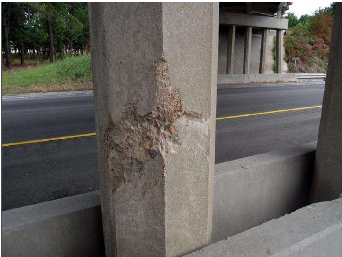
SPALLS IN FACES 1, 2 & 3 OF PILE NO.5 AT BENT 2
