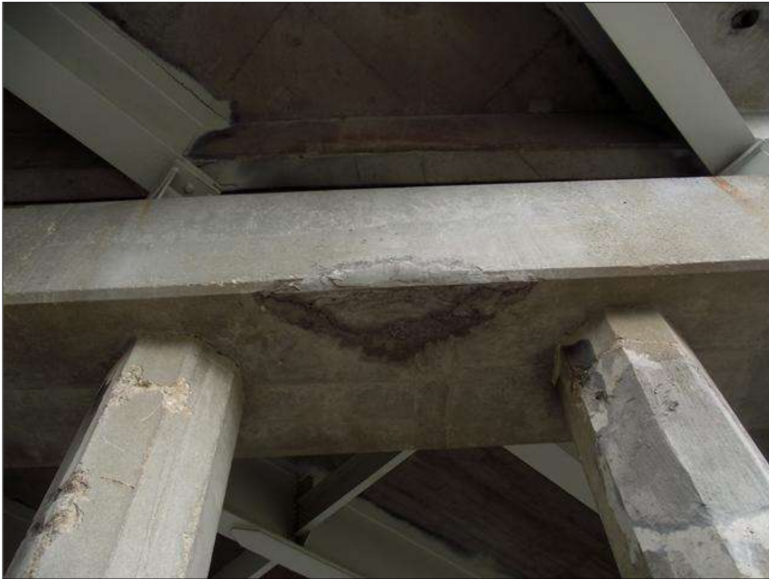
REPAIR PATCH IN THE BOTTOM EDGE OF BENT 2 CAP SPAN 2 SIDE UNDER BAY 3
