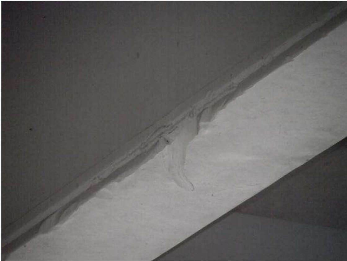
GOUGE IN THE BOTTOM FLANGE OF BEAM 3 IN SPAN 2 AT MIDSPAN
