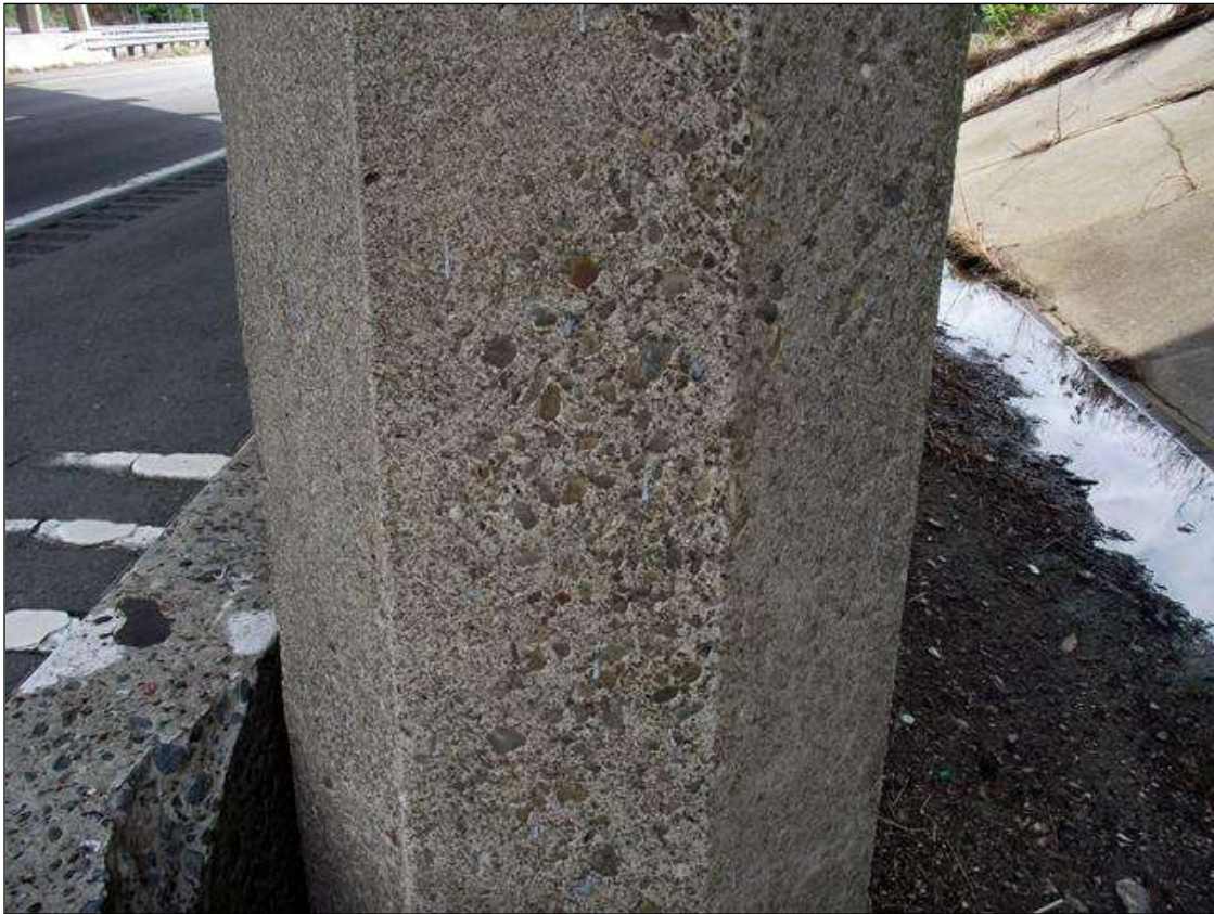
EXTERIOR FACES OF PILES 1 & 7 AT BENT 1 ARE WEATHERED WITH EXPOSED AGGREGATE
