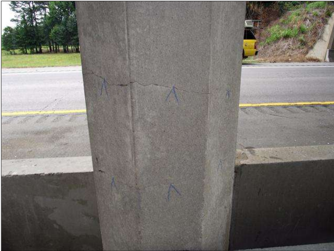
HORIZONTAL CRACKS IN FACES 4, 5, 6, 7 & 8 OF PILE NO.5 AT BENT 2 - PILES 2 & 4 ARE SIMILAR
