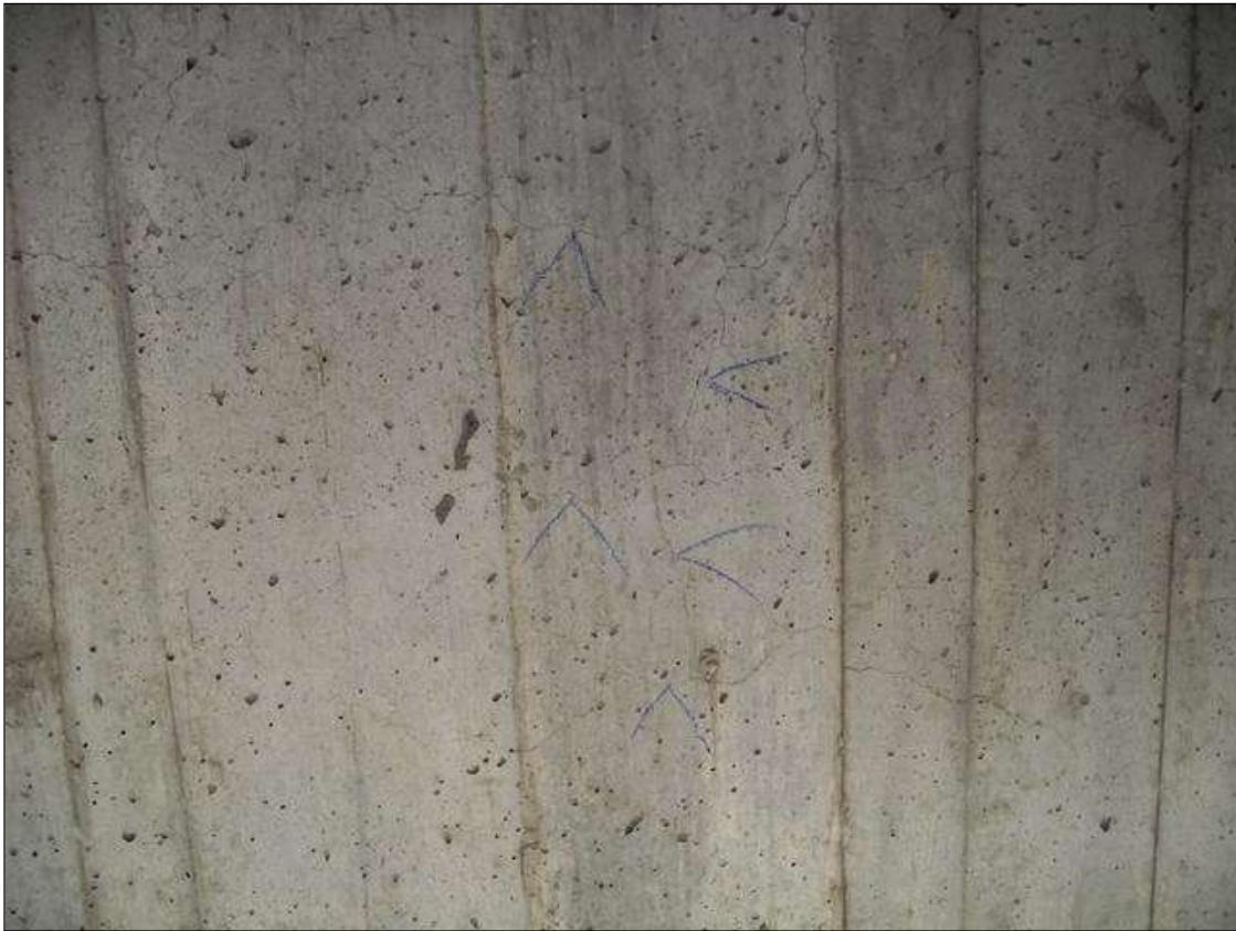
MAP CRACKING ACROSS ORIGINAL BACKWALL AT END BENT 1 BAY 1
