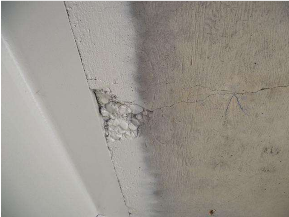
AREA OF HONEYCOMING TO THE LEFT SIDE OF BEAM 2 IN SPAN 1 BAY 1
