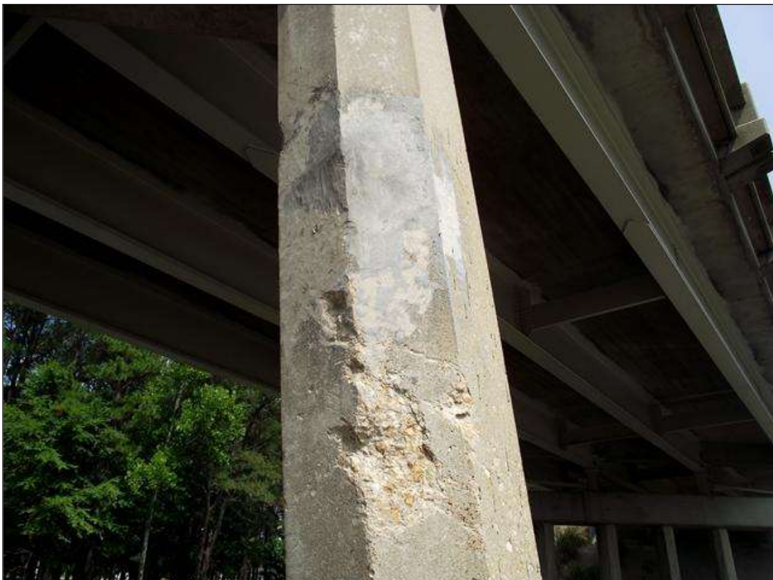
SPALL AND SPALL REPAIR IN FACES 1 & 2 OF PILE NO.7 AT BENT 2
