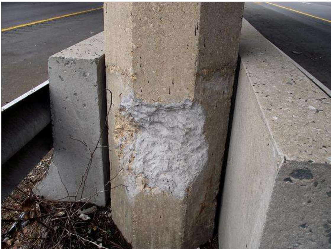
SPALL IN THE RIGHT SIDE OF PILE NO.7 AT BENT 2
