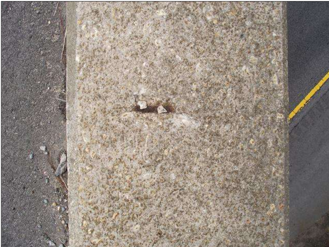
RANDOM SHALLOW SPALLS WITH EXPOSED REBAR ALONG TOP OF CURBLINES
