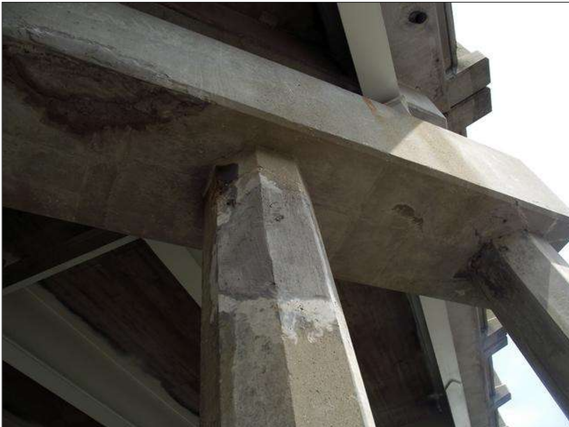
SPALL REPAIR IN FACES 1, 2, 3 & 8 IN PILE NO.6 AT BENT 2
