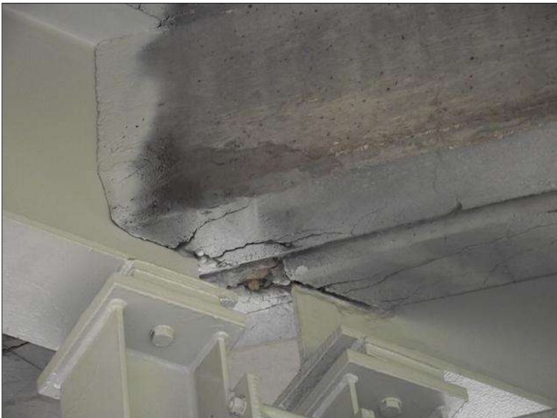
SPAN 3 AND 4 END DIAPHRAGMS AT BENT 3 BAY 2 ARE CRACKED AROUND ENDS OF BEAM 2
