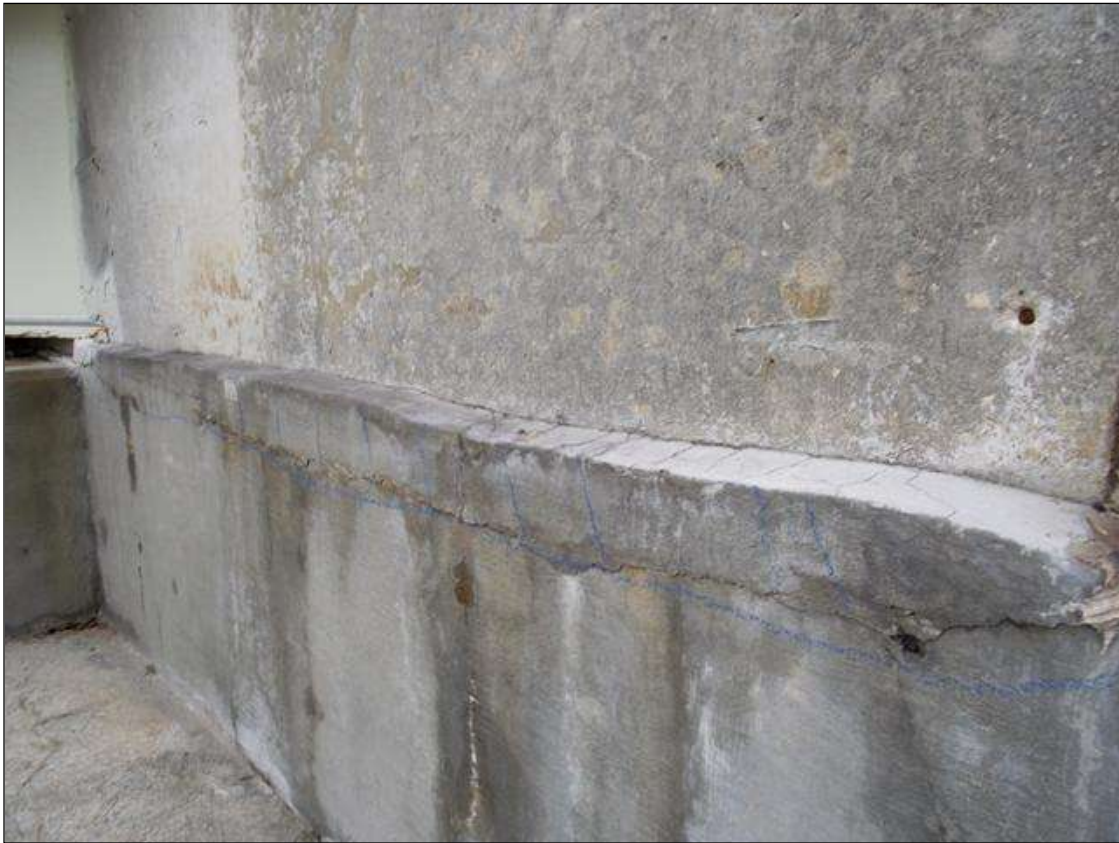
DELAMINATION ALONG TOP EDGE OF BACKWALL ADDITION FROM LEFT END TO BEAM 1 AT END BENT 1
