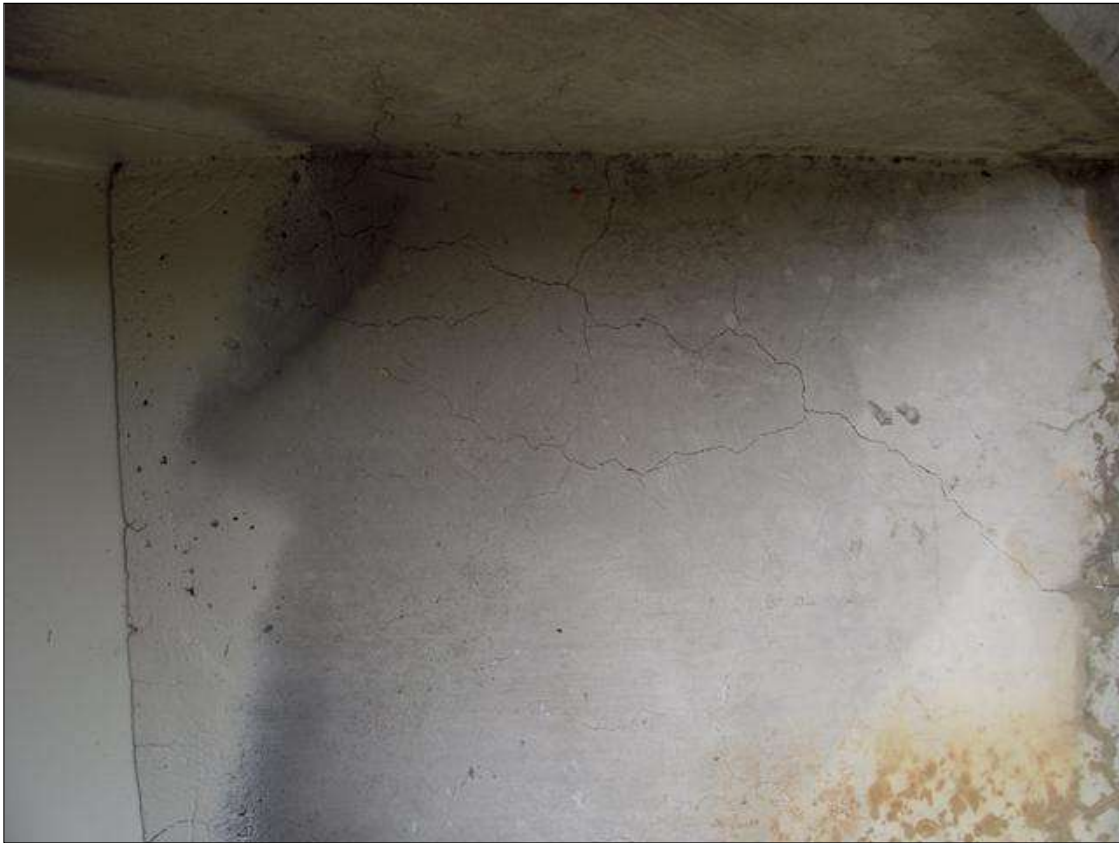
MAP CRACKING IN BACKWALL AT END BENT 2 RIGHT SIDE EXTENSION
