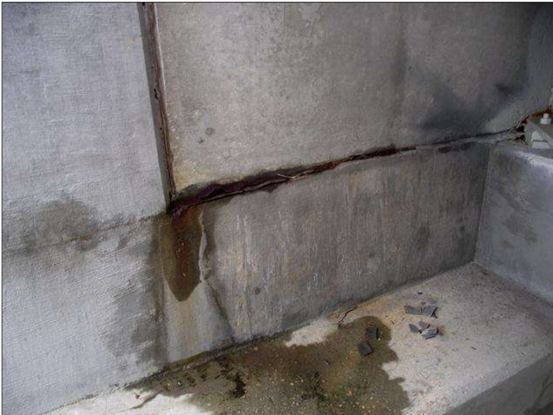
WATER SEEPAGE BETWEEN TOP OF CAP AND NEW PORTION OF BACKWALL AT THE RIGHT SIDE OF END BENT 1
