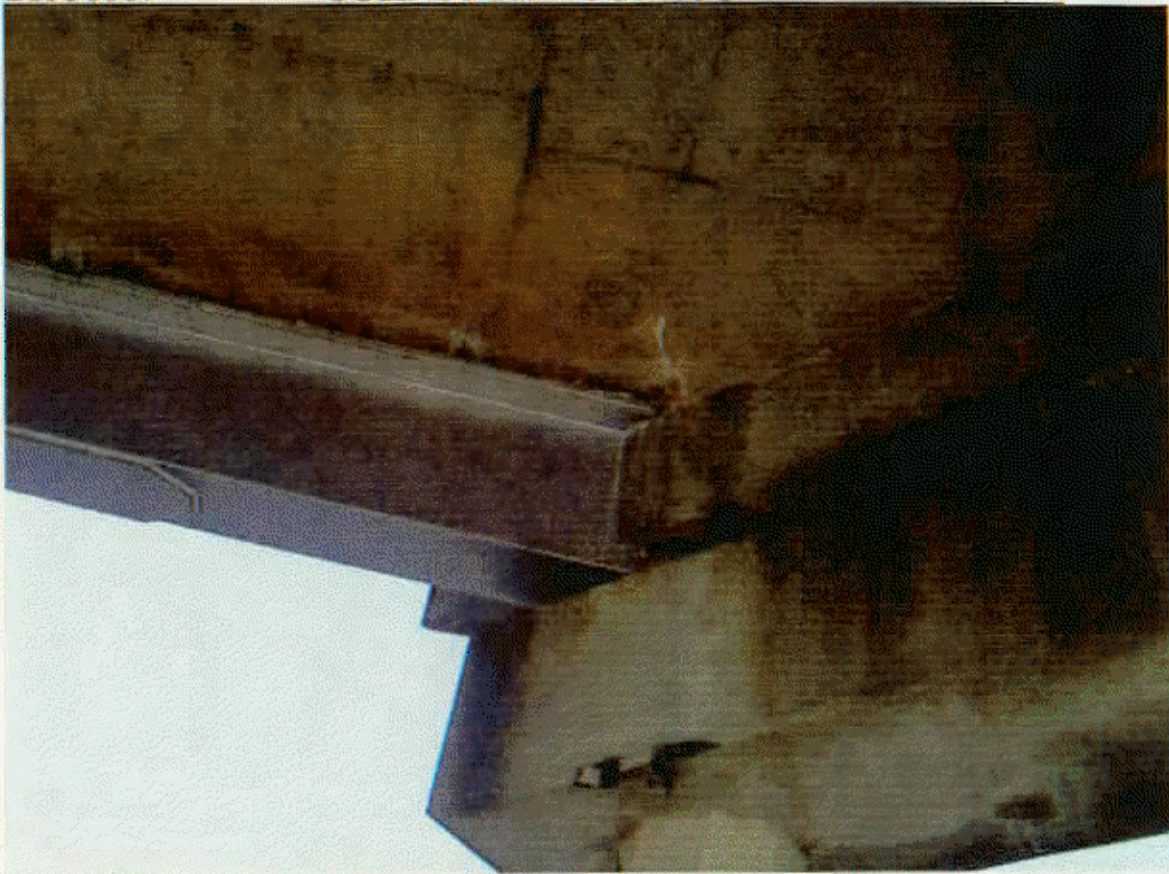
BOTTOM OF DECK HAS DIAG. CR W/ EFFLO AT BT 2 , SP 2 BM 1
