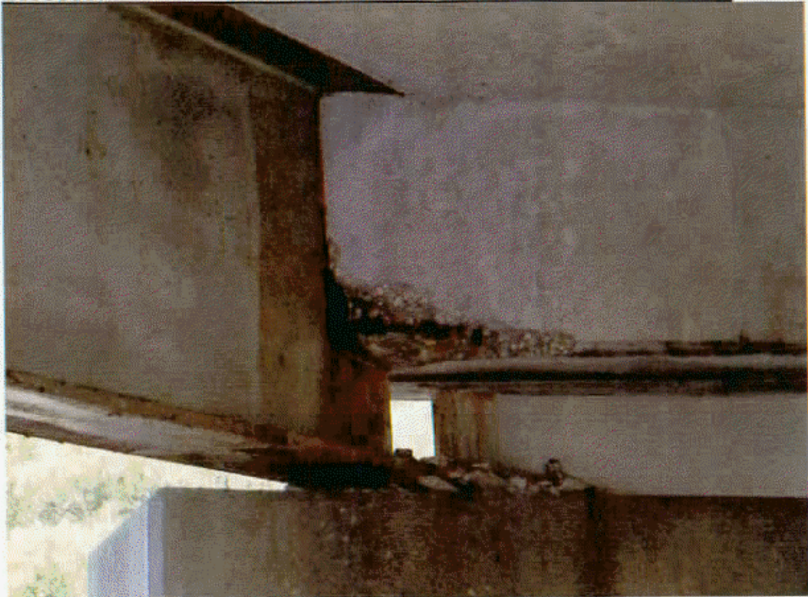
BT 2 SP 1 DIAPH RT OF BM 4 SPALLED W / EXPOSED REBAR
