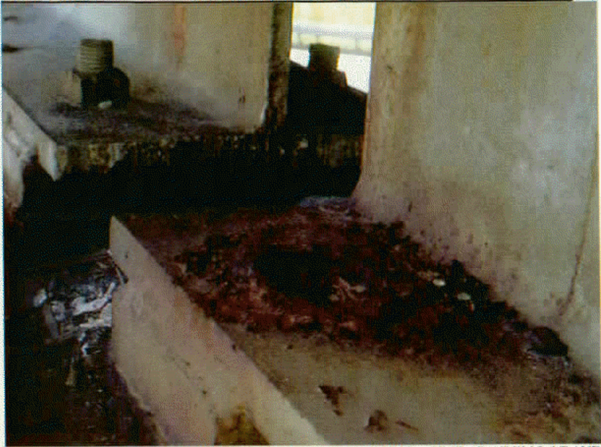
BT 1 SP 1 LT ANCHOR BOLT MISSING, RIGHT IS ALSO MISSING, SIMILAR AT BM 2 LT AND RT. AND ALSO LT SIDE AT BM 3.
