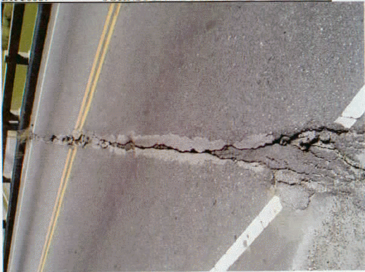
A W S CR W/POTHOLES ALONG JT AT BT 1, SIMILAR AT BTS 2 AND 3
