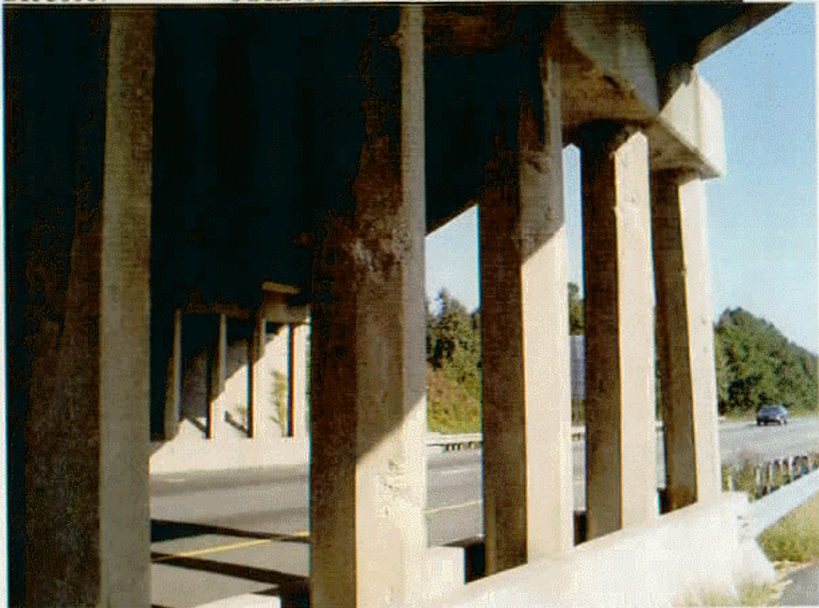
BT 2, P-4 THRU P-7 SPALLED ON SP2 SIDE AND CAP SPALLED W/ REBARS EXPOSED IN BAY 3.
