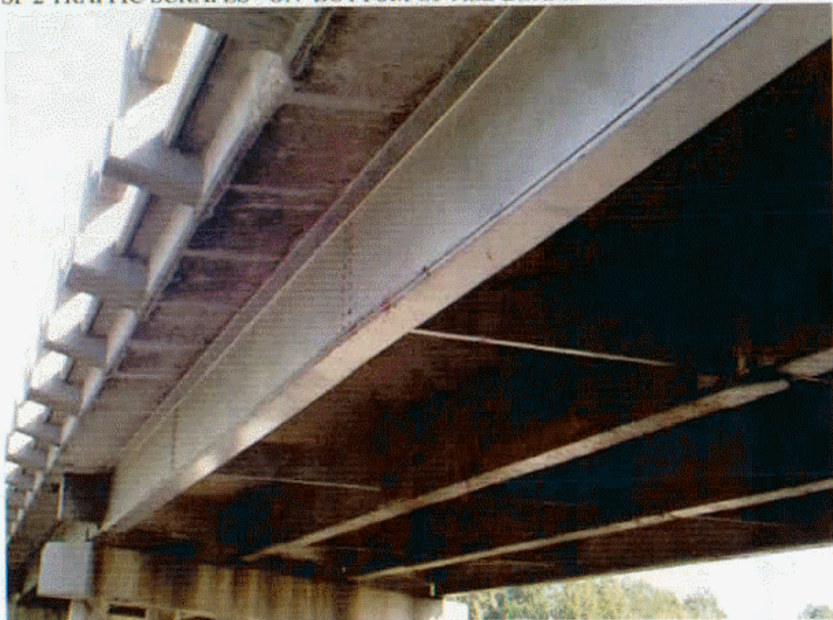
SP 2, BM 1 TRAFFIC DAMAGE HAS CAUSED 2" +/- SWEEP IN BOTTOM FLG AND MINOR SPALLING IN BOTTOM OF OVERHANG
