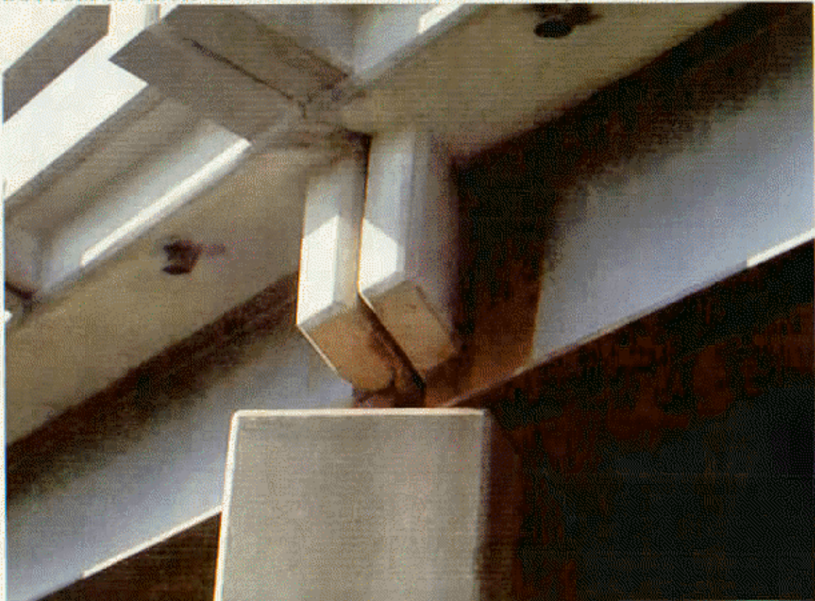
BT 1 , RT END , BMS RUSTING AND RT EXT DIAPH CR AND SPALLING
