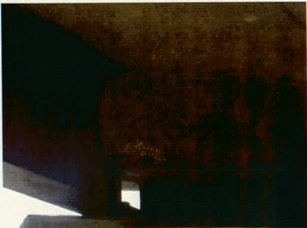
BT 3 SP 4 DIAPH SPALLED LT OF BM 4, SIMILAR AT BM 2
