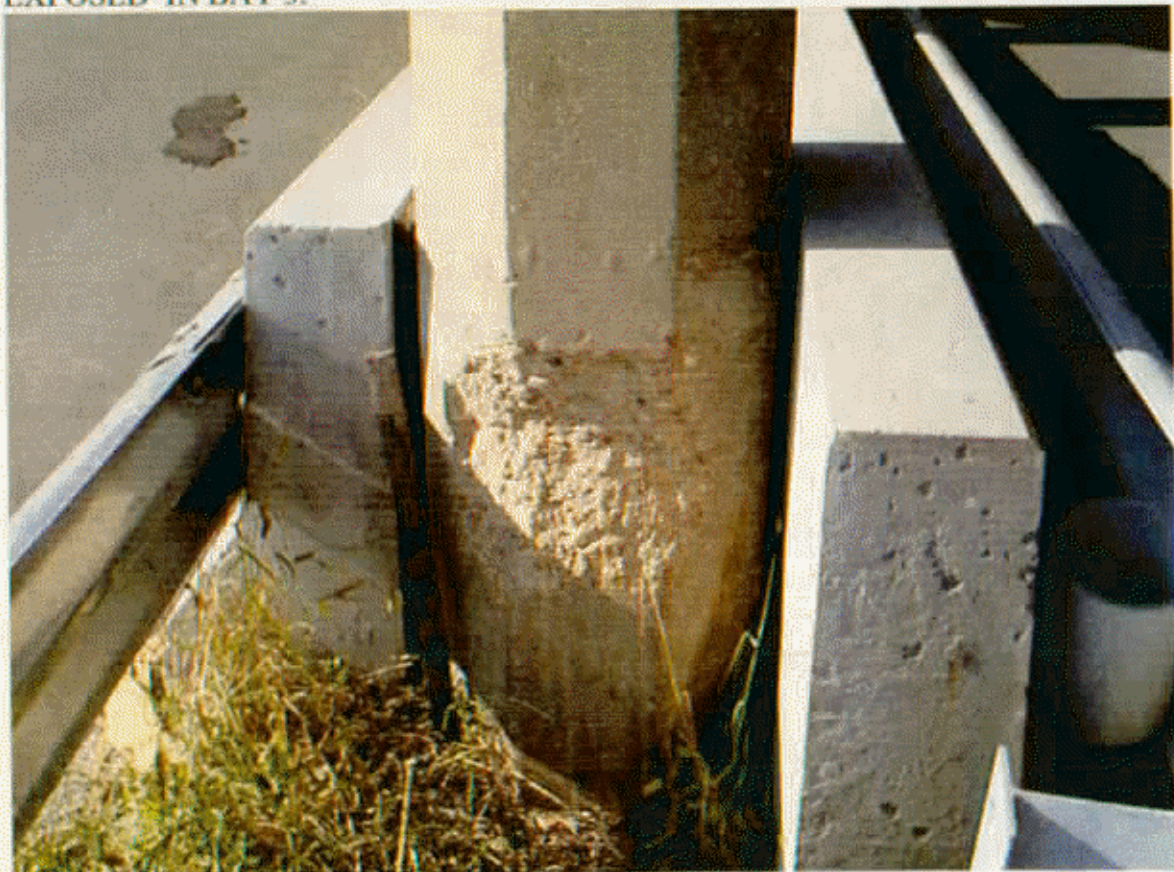
BT 2 P-7 SPALLED IN EAST FACE
