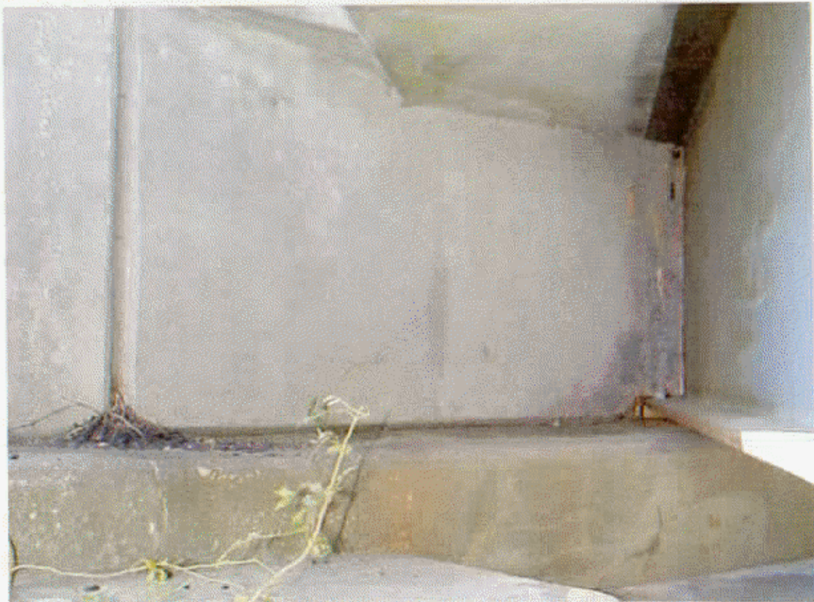
EB 1 RT EXTERIOR CURTAINWALL AND CAP HAVE H/L CRS, SIMILAR AT LT EXTERIOR CURTIANWALL.
