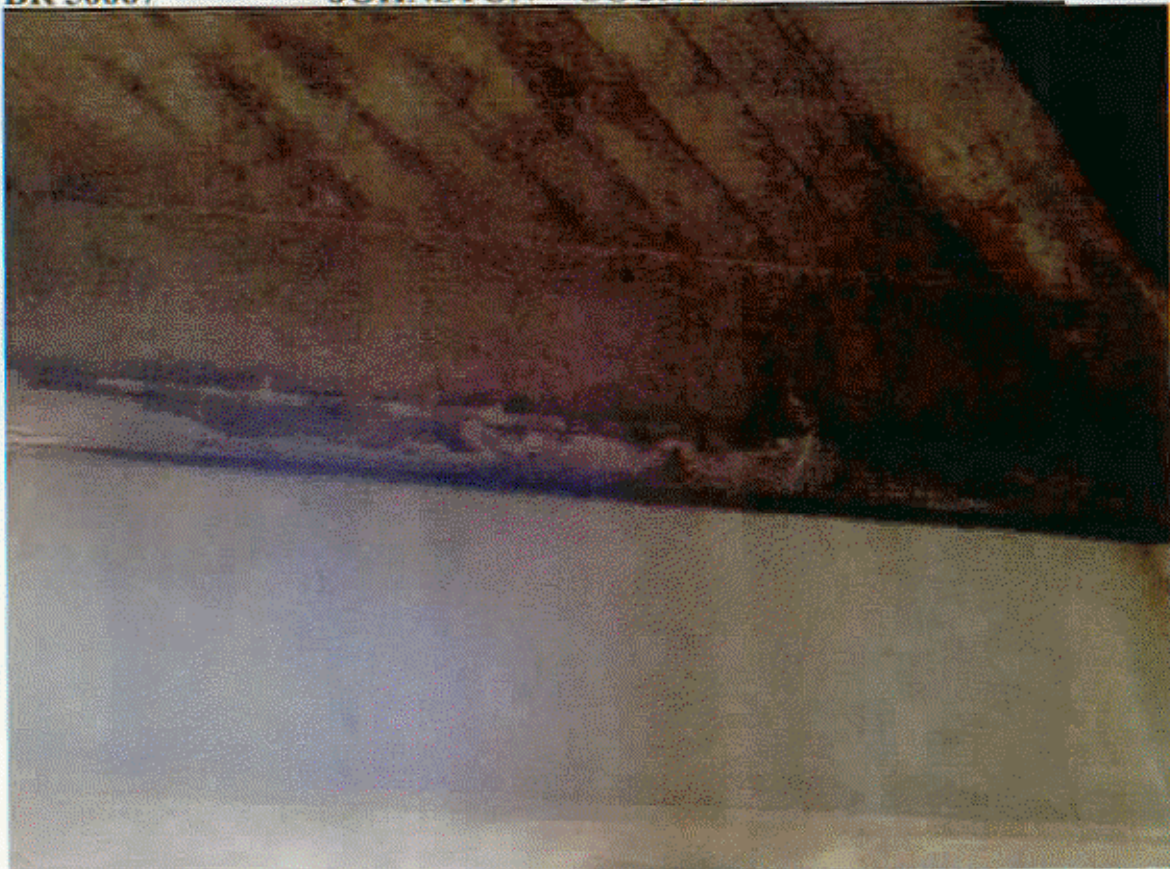
BT 2 SP 3, BAY 3 DIAPH. CR AND SPALLED, SIMILAR CRS IN BAYS 1 AND 2
