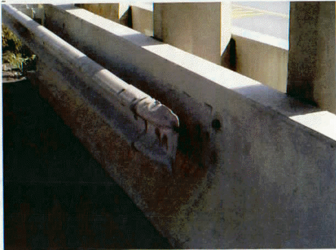
I 95 S.B. LANE GUARDRAIL DETACHED AND STANDING OFF 10" +/-
