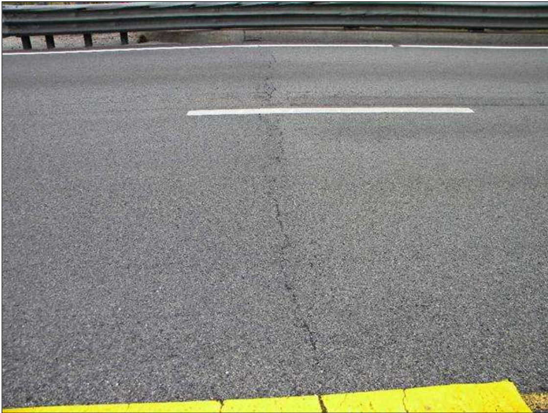
TRANSVERSE CRACK IN WEARING SURFACE OVER END BENT 2
