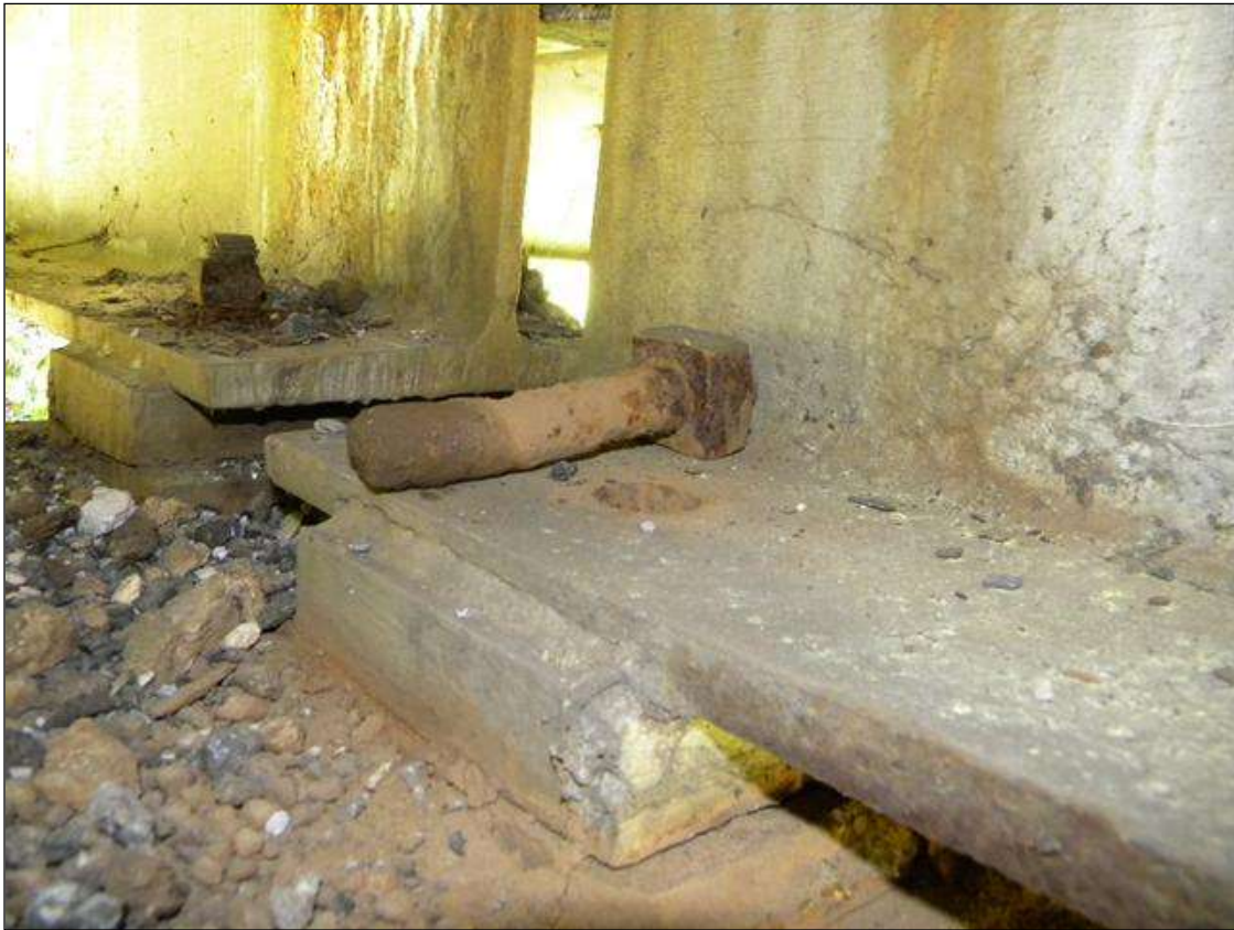
BROKEN ANCHOR BOLT IN THE RIGHT SIDE OF BEAM 2 BEARING ASSEMBLY AT BENT 1 SPAN 2 (PRIORITY MAINTENACNE ISSUED)
