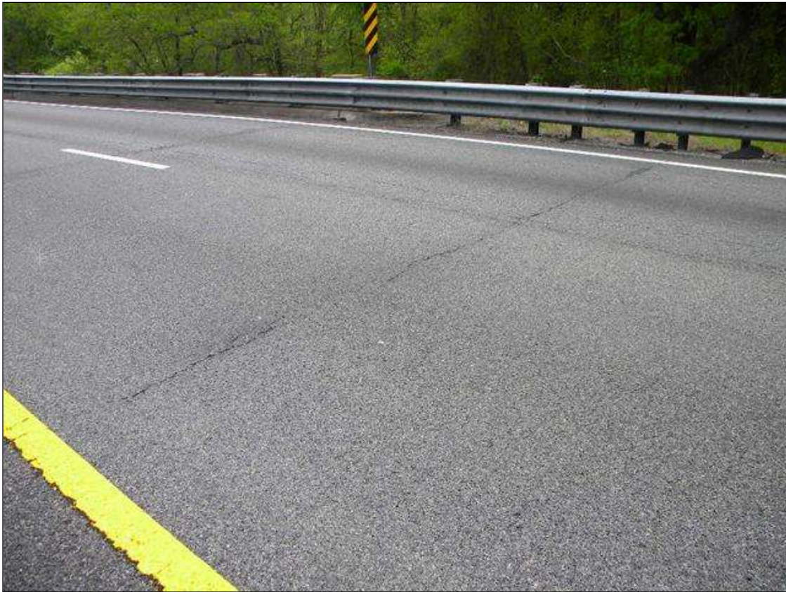
TRANSVERSE CRACK IN APPROACH 1
