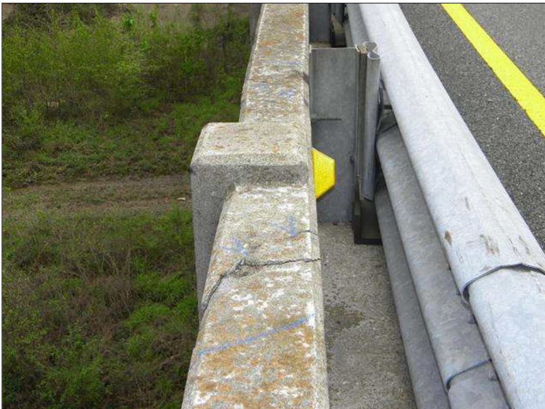
LEFT SIDE GUARDRAIL IN SPAN 2 IS CRACKED AND SPALLING FROM IMPACT DAMAGE
