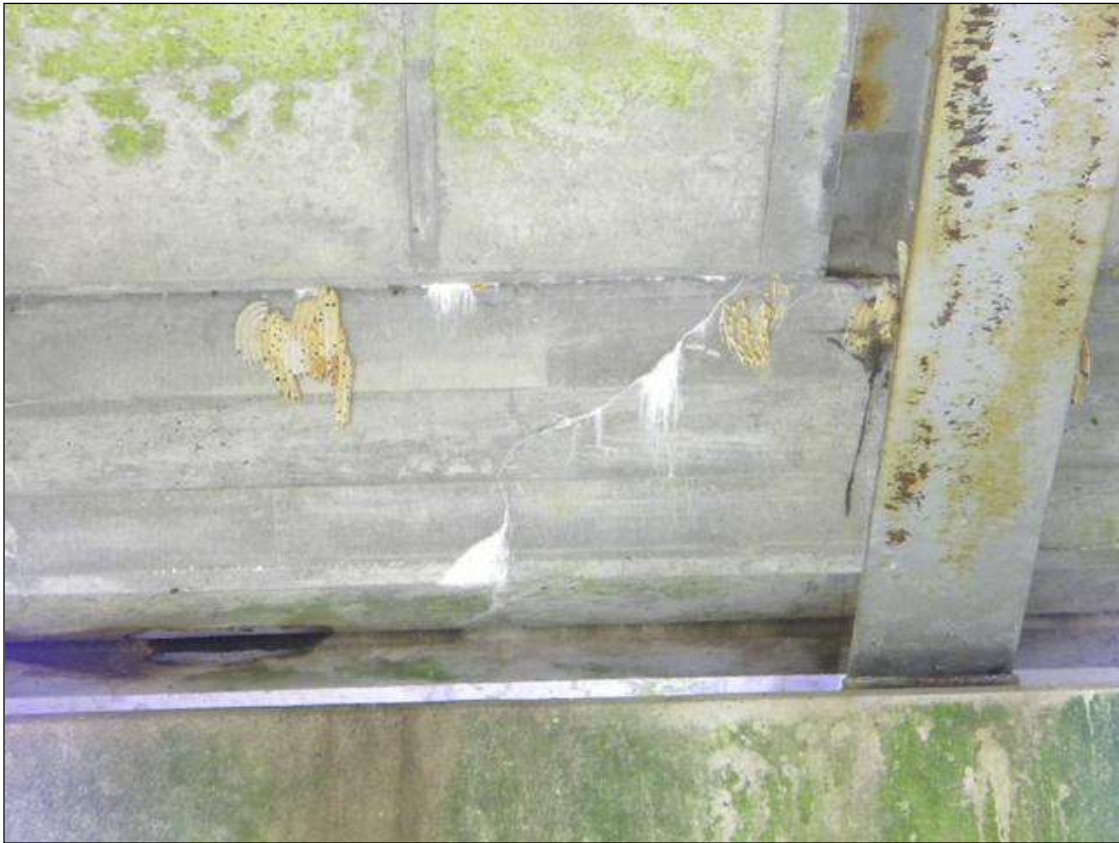
HAIRLINE VERTICAL AND DIAGONAL CRACKS WITH EFFLORESCENCE IN SPAN 3 END DIAPHRAGM AT BENT 2
