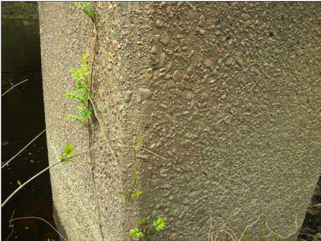
BENT COLUMNS SCALED WITH COARSE AGGREGATE EXPOSED UP TO HIGH WATERMARK
