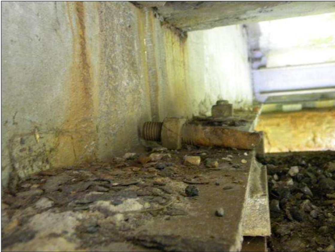
BROKEN ANCHOR BOLT IN THE LEFT SIDE OF BEAM 3 BEARING ASSEMBLY AT BENT 1 SPAN 2 (PRIORITY MAINTENACNE ISSUED)
