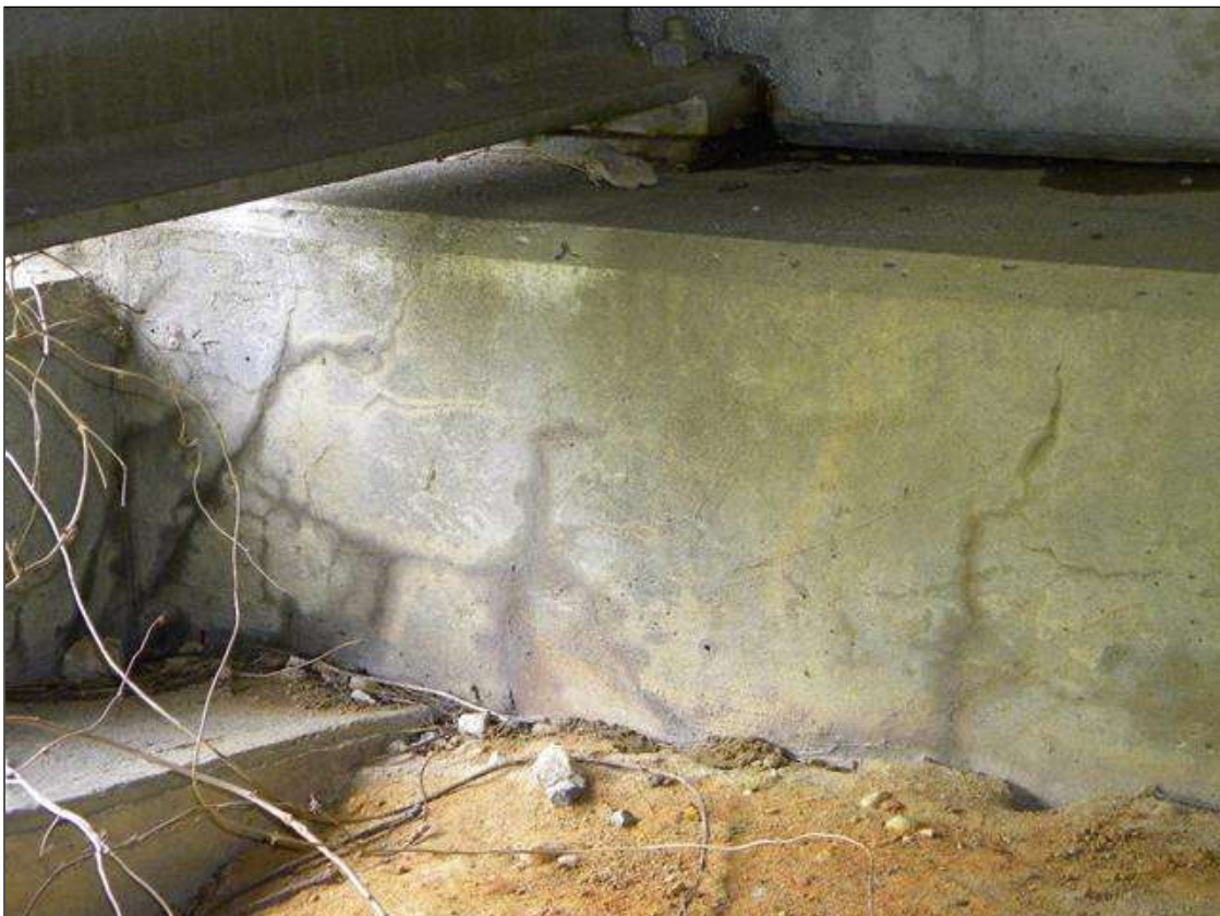
HAIRLINE MAP CRACKING IN FACE OF CAP AT END BENT 2 UNDER BEAM 1
