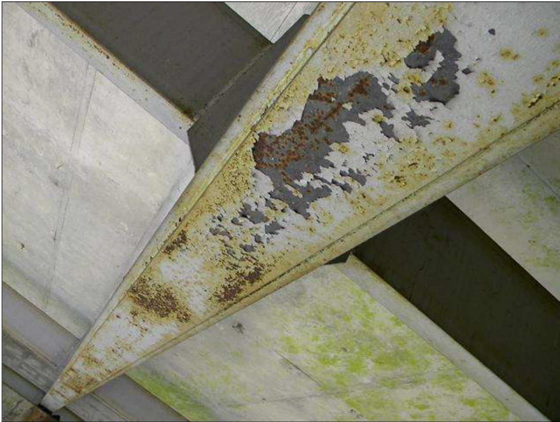
PEELING PAINT & SURFACE RUST IN THE BOTTOM OF COVER PLATES FOR BEAMS 2 & 3 IN SPAN 4
