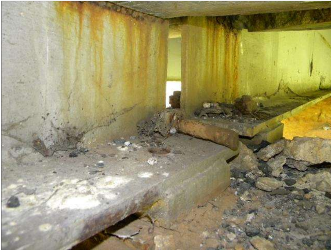
BROKEN ANCHOR BOLT IN THE LEFT SIDE OF BEAM 2 BEARING ASSEMBLY AT BENT 1 SPAN 2 (PRIORITY MAINTENACNE ISSUED)
