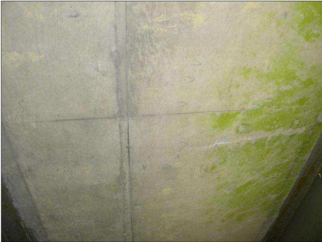
HAIRLINE LONGITUDINAL AND TRANSVERSE CRACKS IN BOTTOM OF DECK OF SPAN 4
