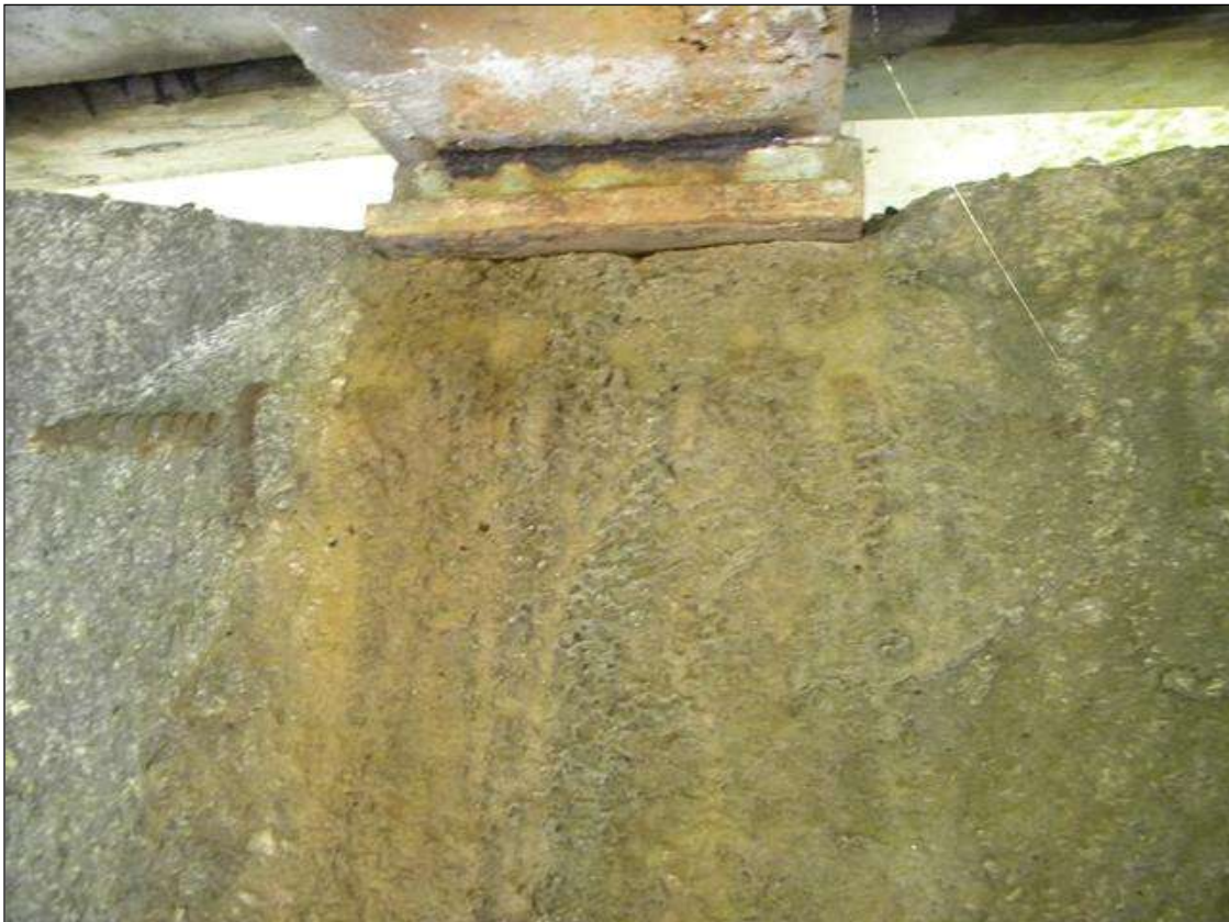
SPALL IN BENT 1 CAP SPAN 2 SIDE AT BEAM 3, PHOTO 1 OF 2 (PRIORITY MAINTENACNE ISSUED)
