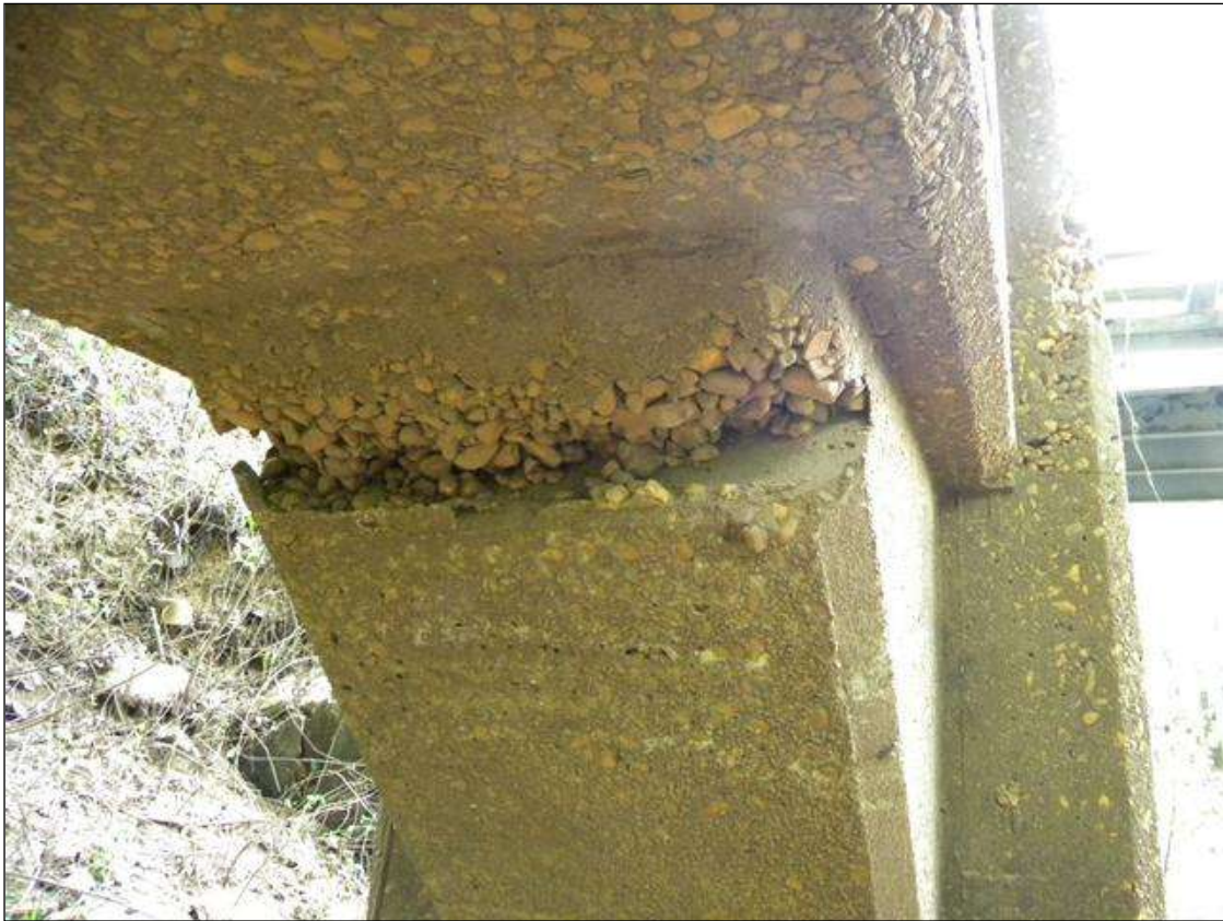
HONEYCOMBED AREA IN THE LOWER FILLET OF COLUMN 1 AT BENT 1
