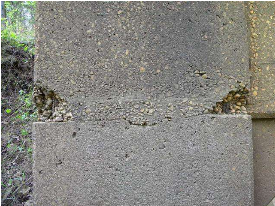
TWO "HONEYCOMBED" AREAS WITH EXPOSED REBAR IN COLUMN 2 AT BENT 1 SPAN 2 SIDE
