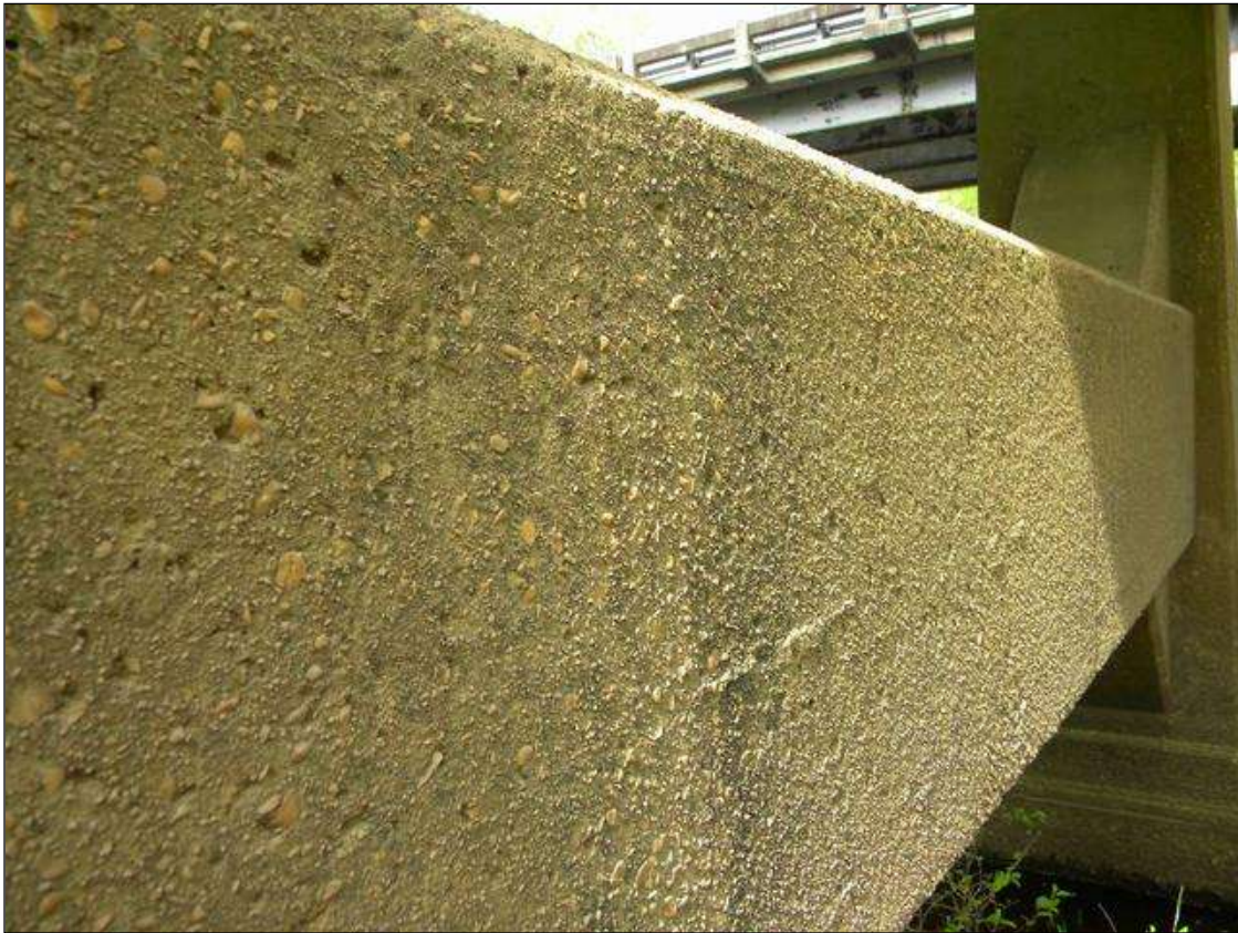
BENT STRUTS SCALED WITH COARSE AGGREGATE EXPOSED
