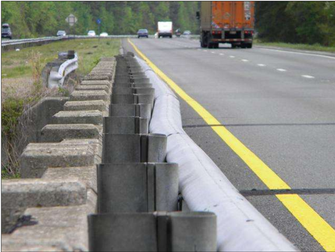
IMPACT DAMAGE ALONG THE LEFT SIDE STEEL GUARDRAIL OF SPAN 2
