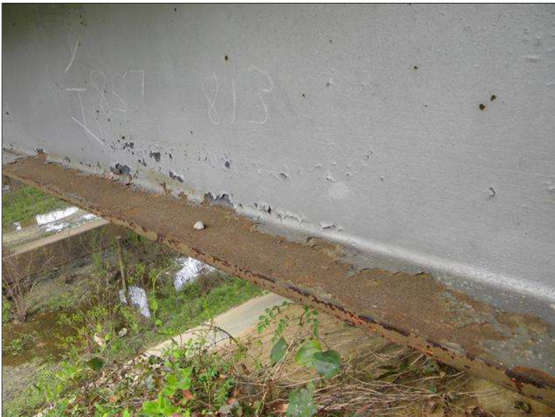
PEELING PAINT & SURFACE RUST IN THE RIGHT SIDE BOTTOM FLANGE OF BEAM 4 IN SPAN 4 OUT 10 FT. FROM END BENT 2
