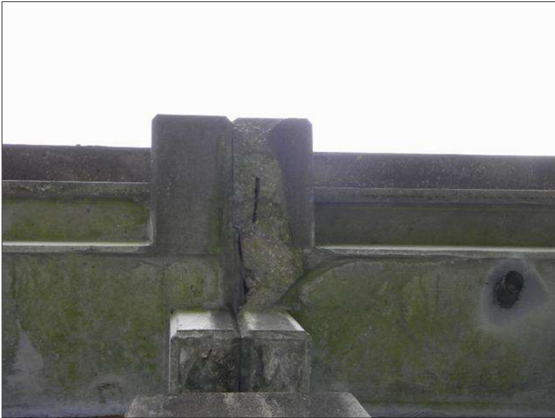
SPALLING WITH EXPOSED REBAR IN GUARDRAIL END POST BASE AT THE LEFT SIDE OF BENT 3 SPAN 3 SIDE
