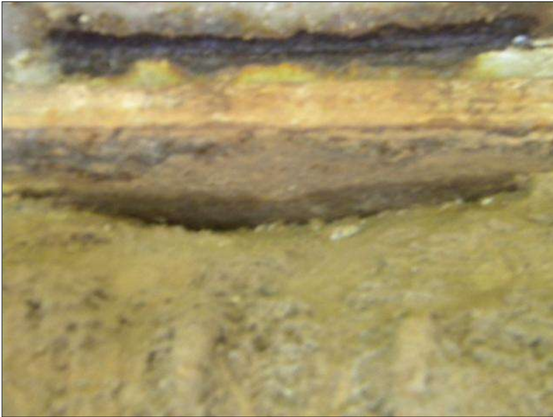
LAREG SPALL WITH EXPOSED MASONRY PLATE AT BEAM 3 BENT 1 SPAN 2 SIDE, PHOTO 2 OF 2 (PRIORITY MAINTENACNE ISSUED)
