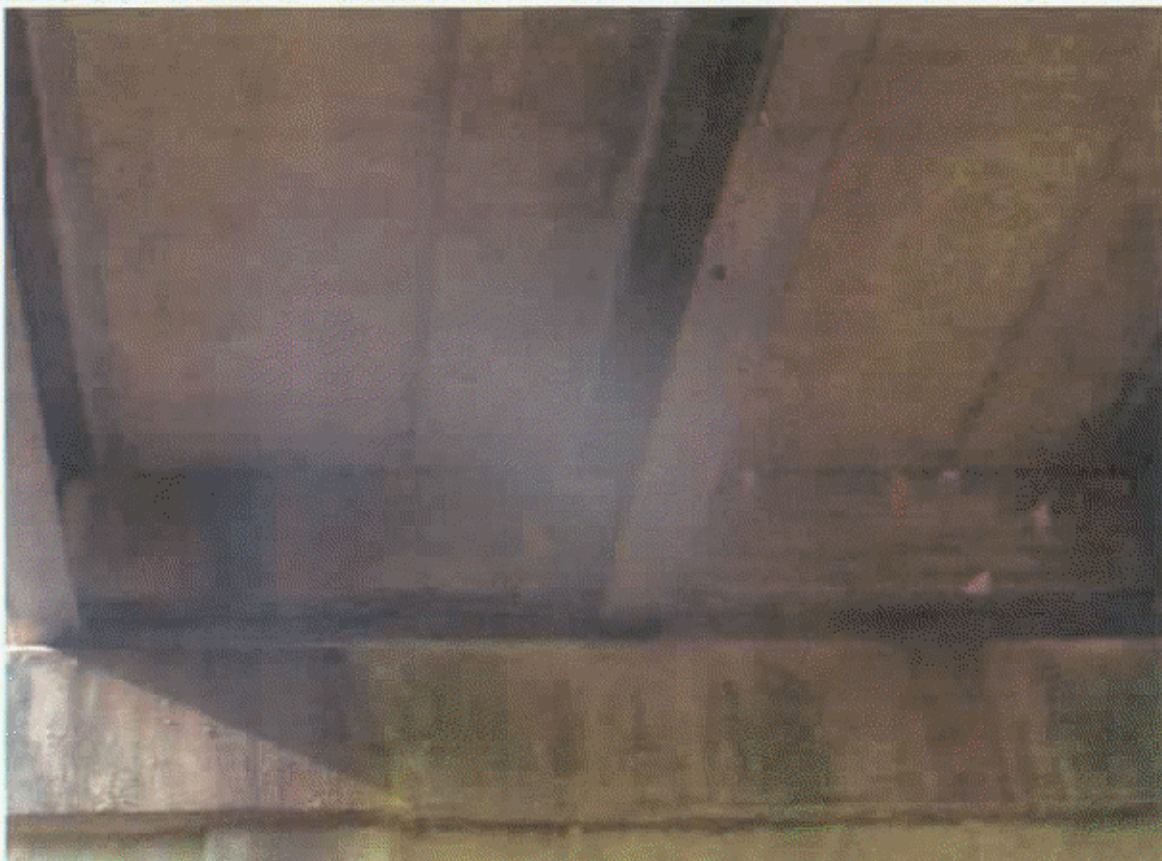
BAY 2, & 3 SPAN 3 AT BENT 2 EFFLO. CRACKS & LEAKS @ DECK
