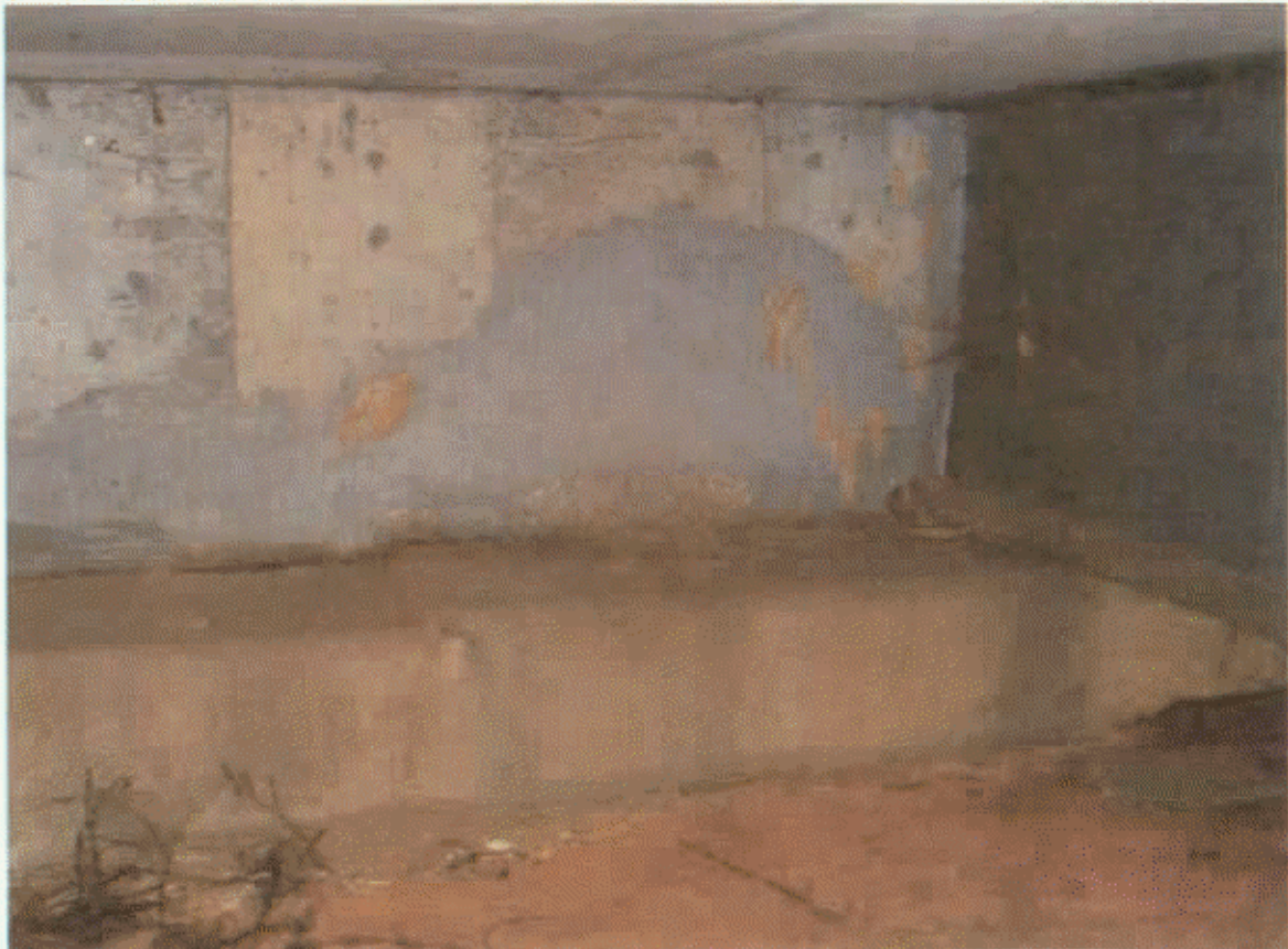
BAY 3 AT END BENT 1 CURTAINWALL SPALLS AND LEAKAGE
