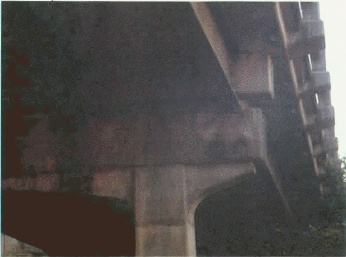
BENT 1 CAP AT BEAM 1 SPAN 2 SPALLED (P.A.)
