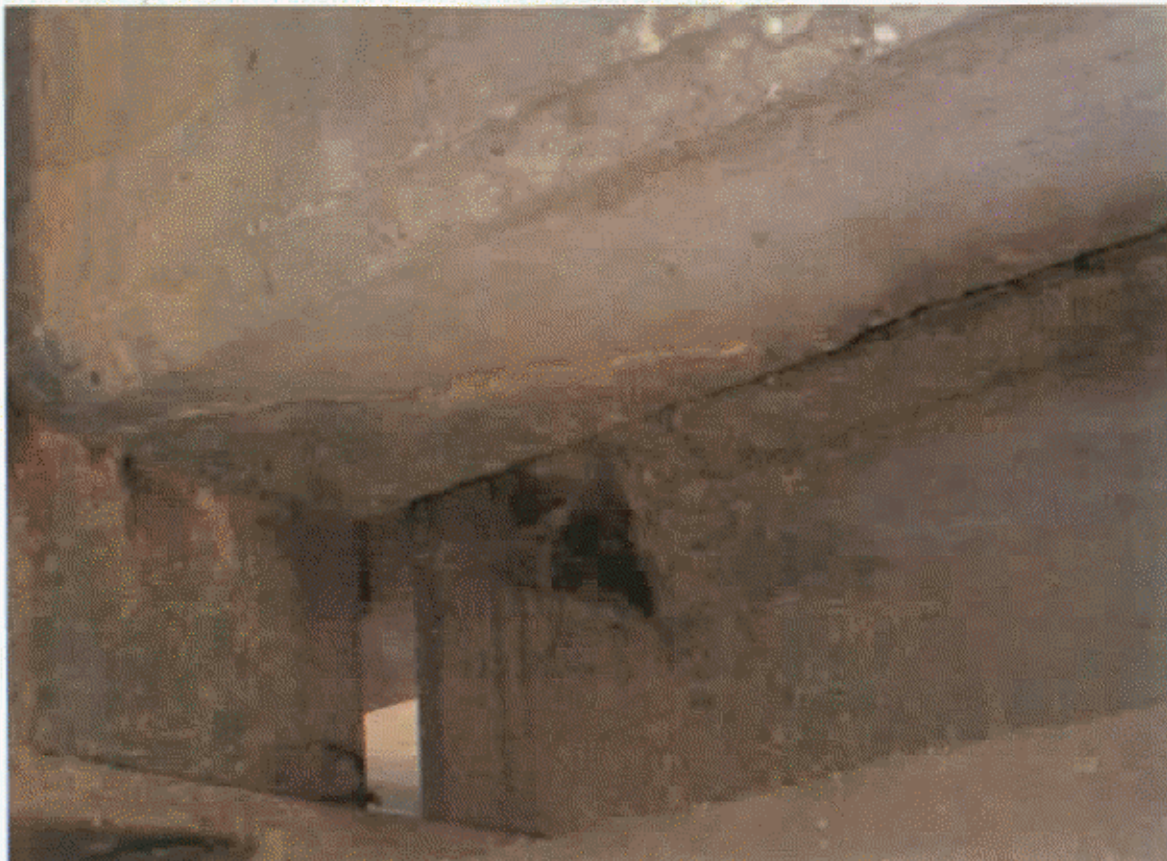
BY. 3 DIAPHRAGM SP. 1, & 2 AT BT. 1 SPALLS @ EXTERIOR JOINT
