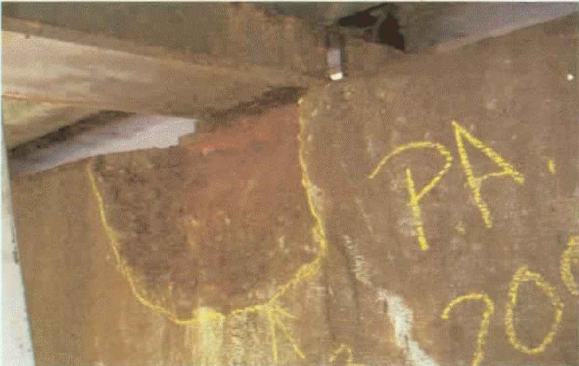
BENT 1 CAP AT BEAM 3, SPAN 1 SPALLED AT EAST ANCHOR BOLT 20"W X 13"H X 10"D (P.A.)
