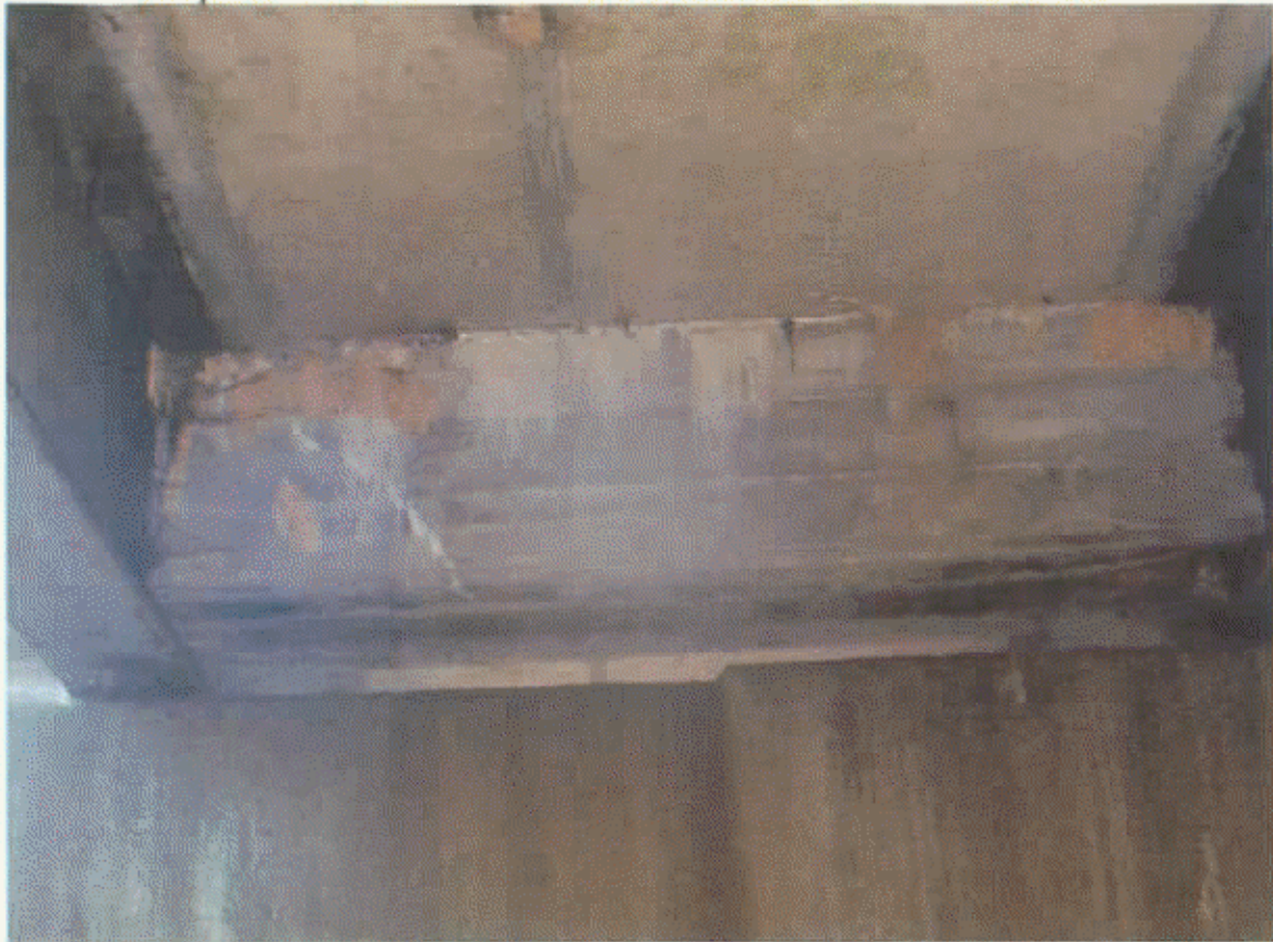
END DIAPHRAGM IN BAY 1, SPAN 1 AT BENT 1 CRACKED /EFFLO
