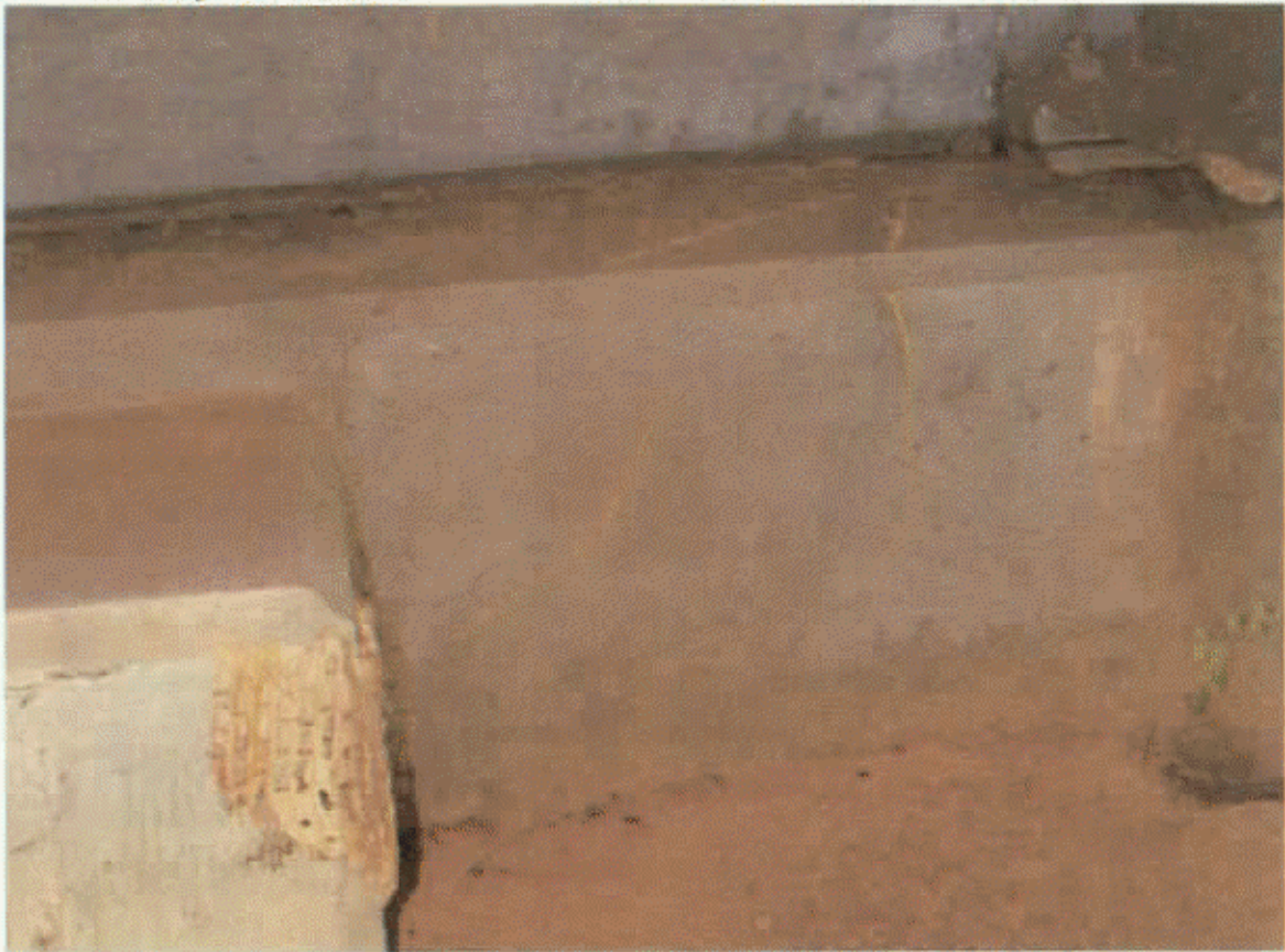
END BENT 2 CAP AT BRACE PILE 2 WITH DIAGONAL CRACK
