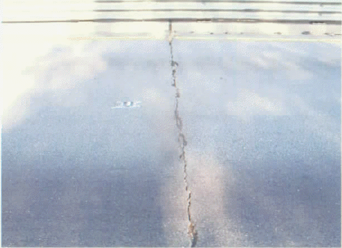
ASPHALT WEARING SURFACE AT BENT 1 JOINT
