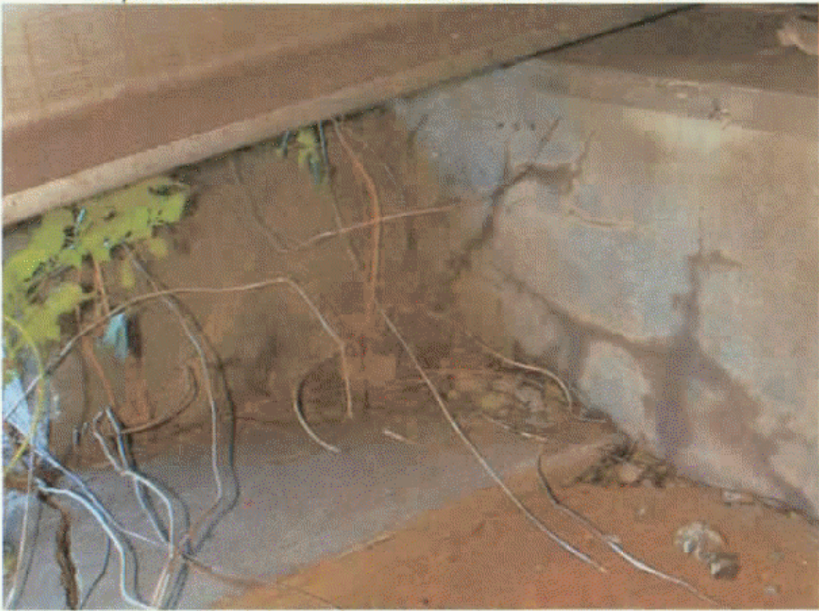
END BENT 2 MAPCRACKS AT BRACE PILE 3
