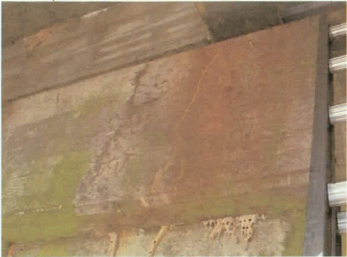
BENT 3 CAP SPAN 4 SIDE AT BEAM 3 CAP CRACKS
