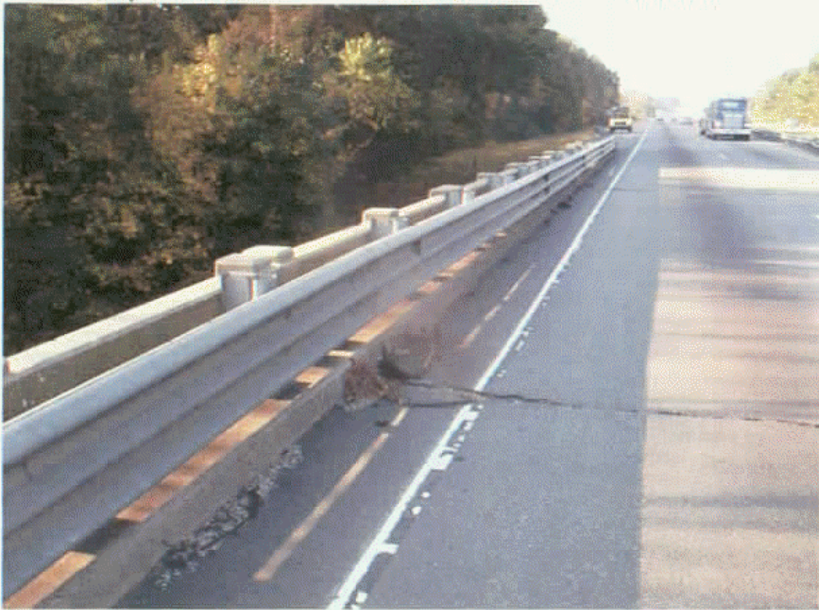
DEBRIS ALONG EAST CURB
