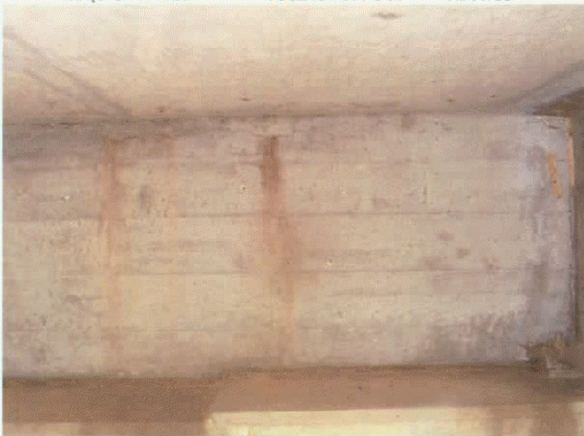
BAY 3 END BENT 2 CURTAINWALL W/ HORIZ. CRACKS 2" DOWN
