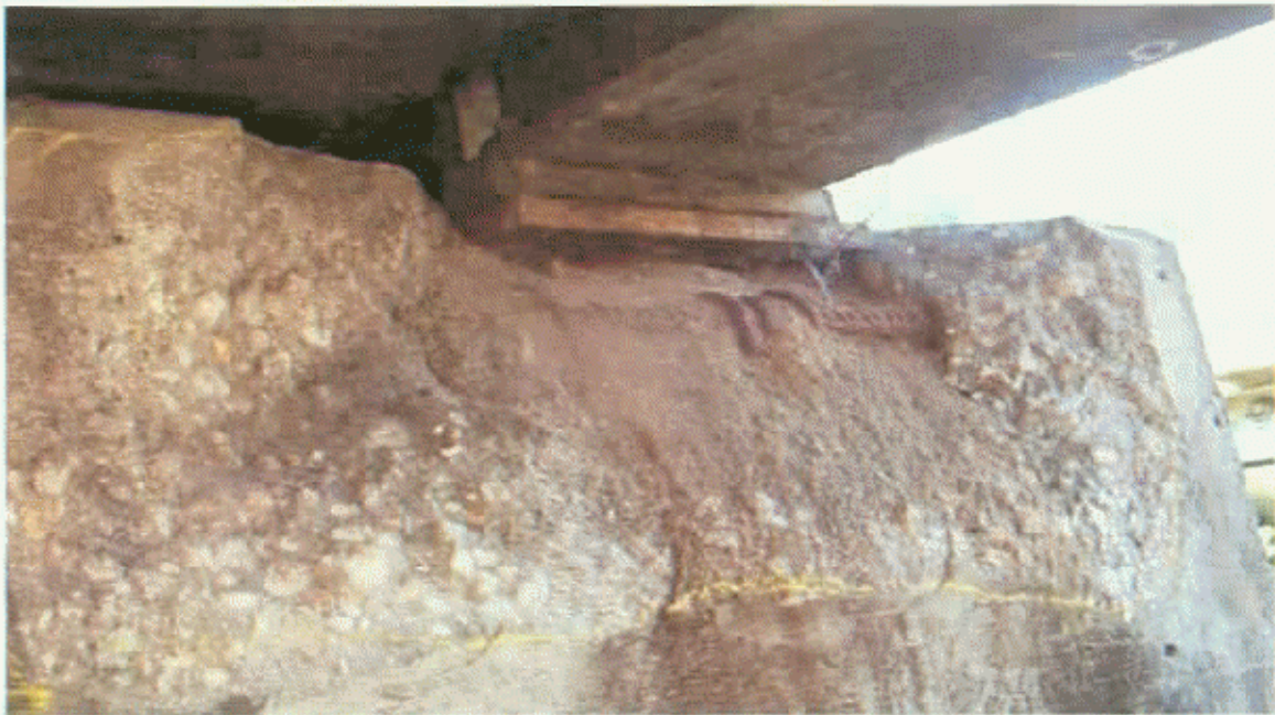
BENT 1 CAP AT BEAM 1 OF SPAN 2 SPALLED 15" X 34" X 10 1/2" 1" BEYOND ANCHOR BOLTS (P.A.)
