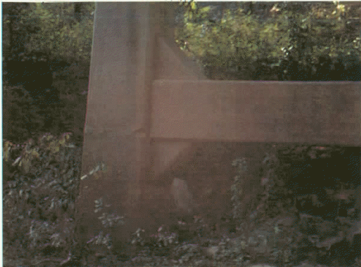
COLUMN 2, AT BENT 1 MINOR HONEYCOMB
