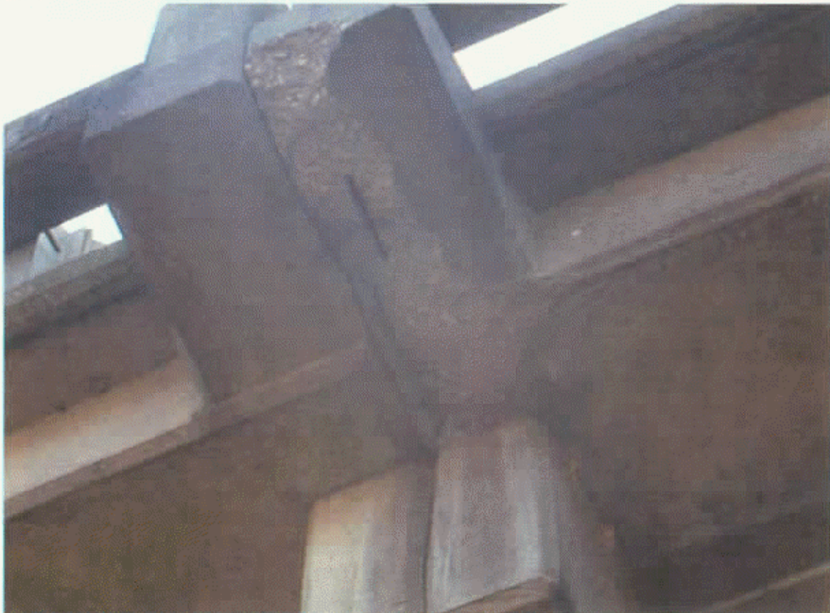
WEST RAIL AT BENT 3 UNDERSIDE SPALLED
