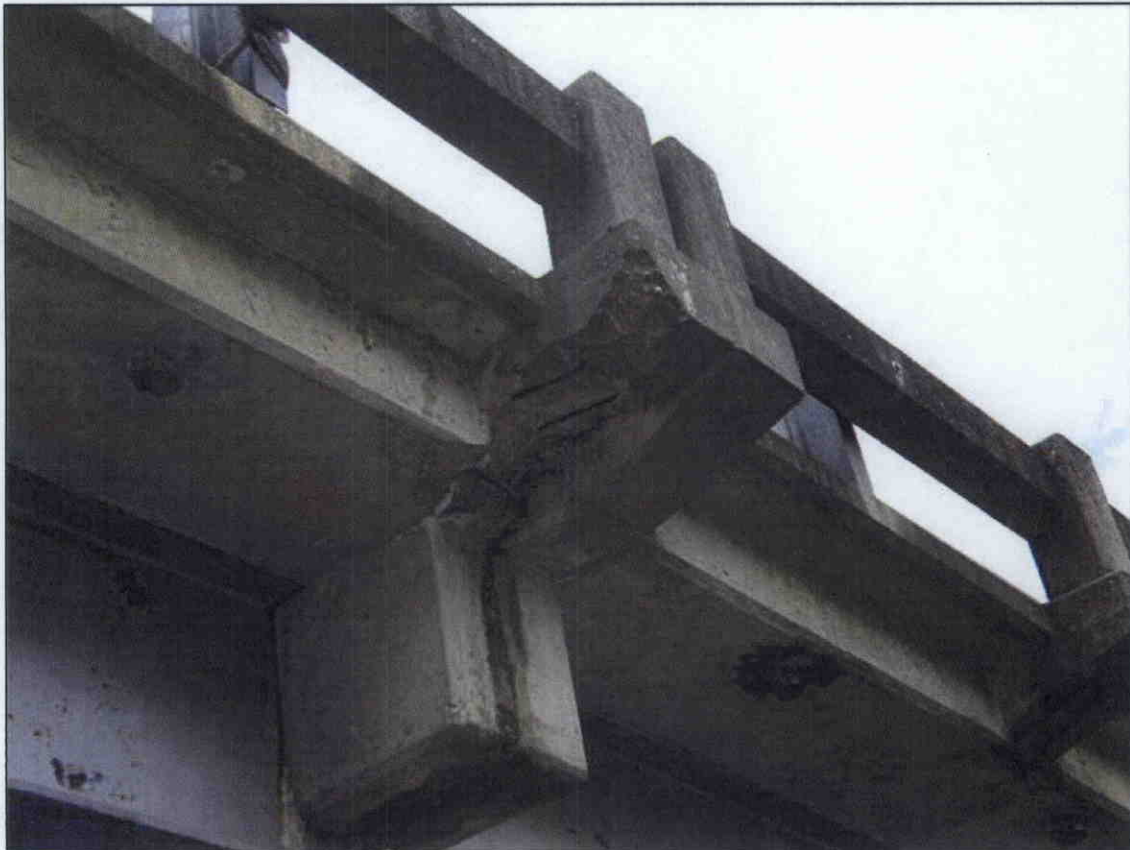
GUARDRAIL END POST BASE AT THE RIGHT SIDE OF BENT 1 SPAN 1 SIDE IS SPALLED WITH EXPOSED REBAR
