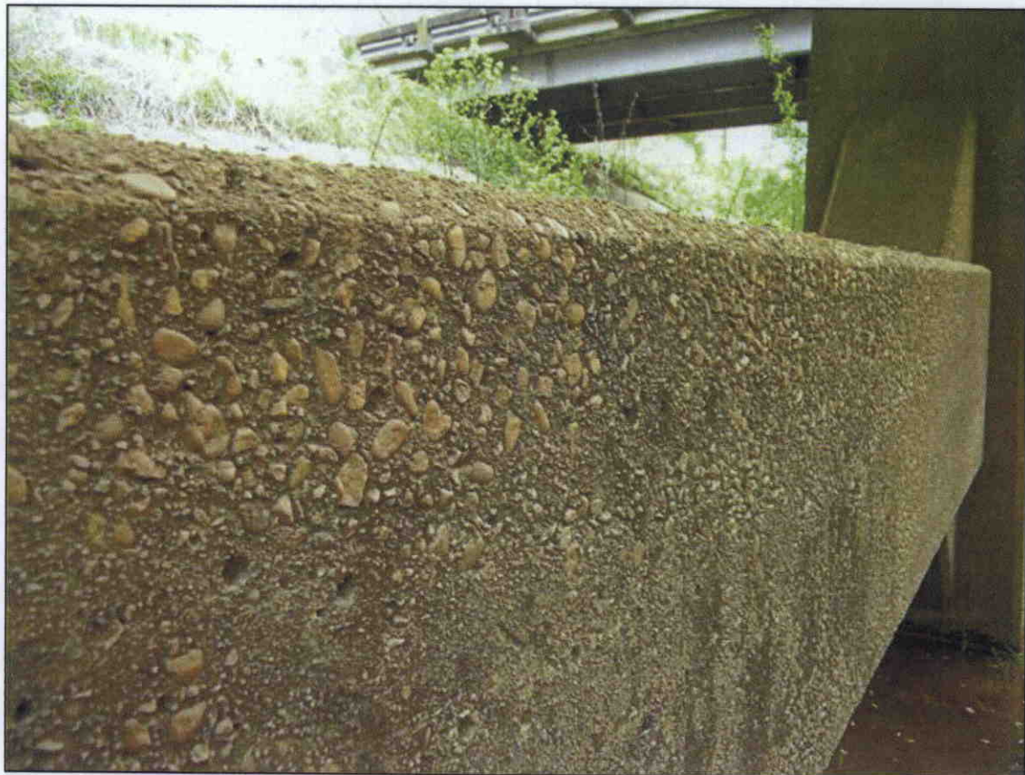
BENT STRUTS SCALED WITH COARSE AGGREGATE EXPOSED
