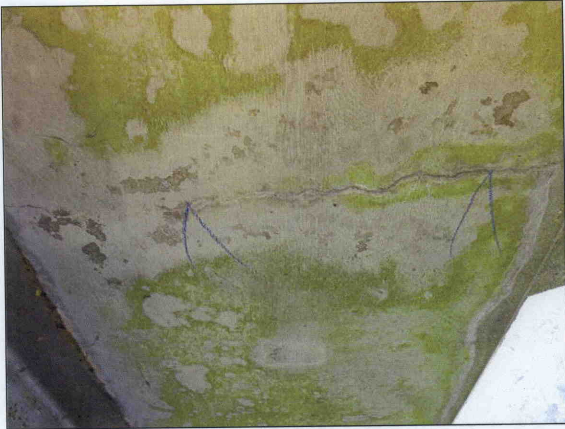
RANDOM HAIRLINE TRANSVERSE CRACKS WITH EFFLORESCENCE IN DECK OVERHANGS
