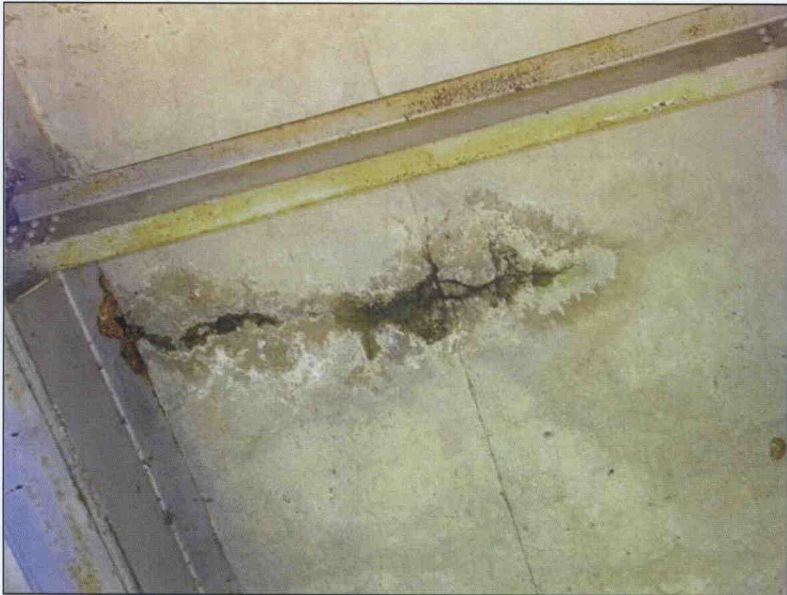
TRANSVERSE CRACK WITH WATER SEEPAGE IN BOTTOM OF DECK SPAN 3 BAY 2 AT 1/3 POINT FROM BENT 2
