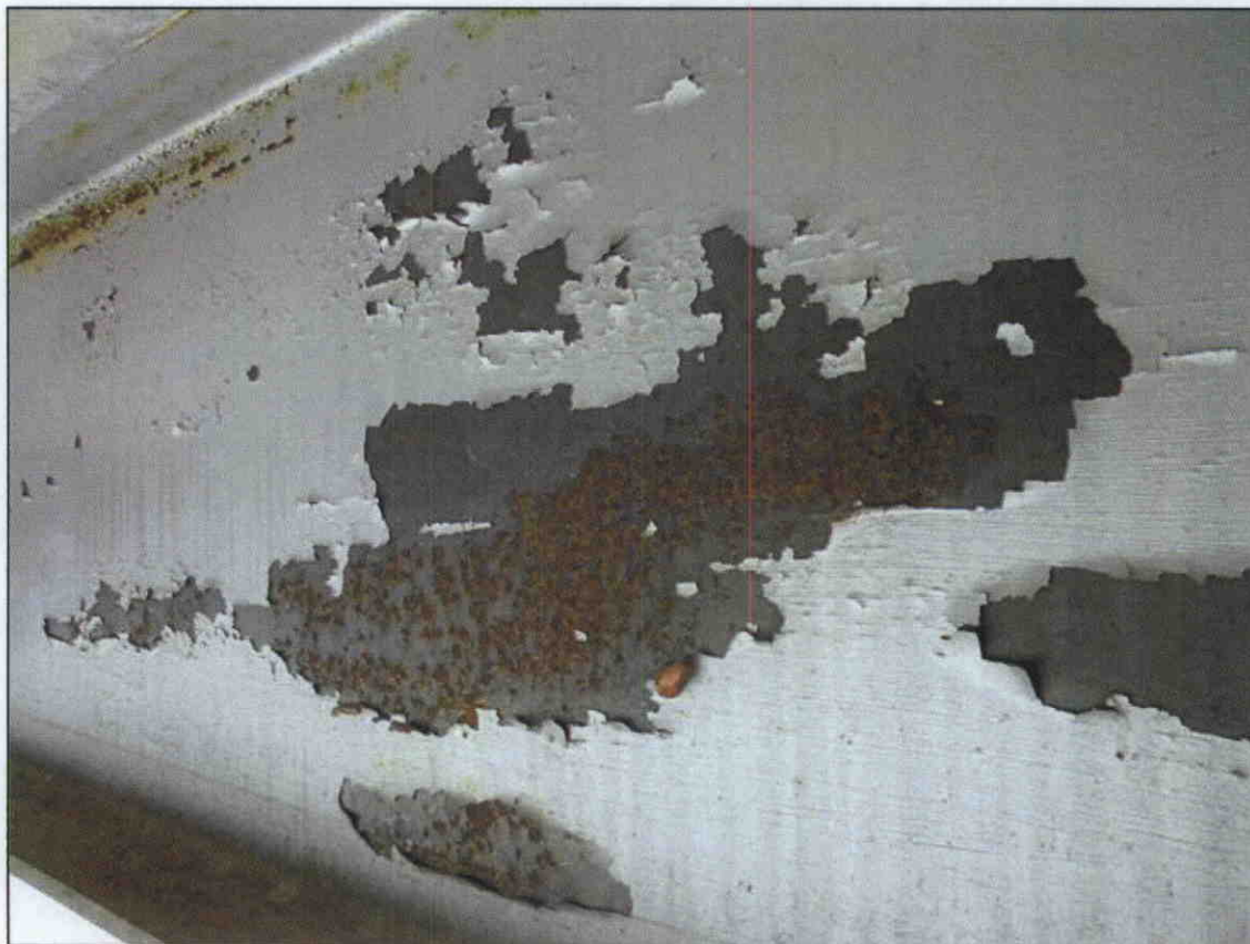
RANDOM SPOTS OF PEELING PAINT AND SURFACE RUST IN BEAM WEBS
