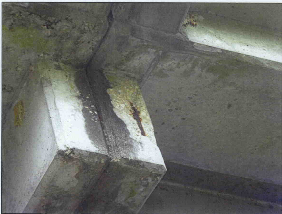
SPALL WITH EXPOSED REBAR IN LEFT EXTERIOR DIAPHRAGM AT BENT 2 SPAN 2 SIDE
