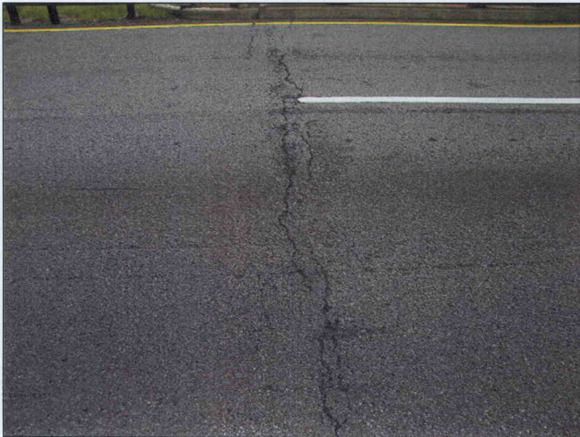
TRANSVERSE CRACKS IN WEARING SURFACE OVER END BENT 2
