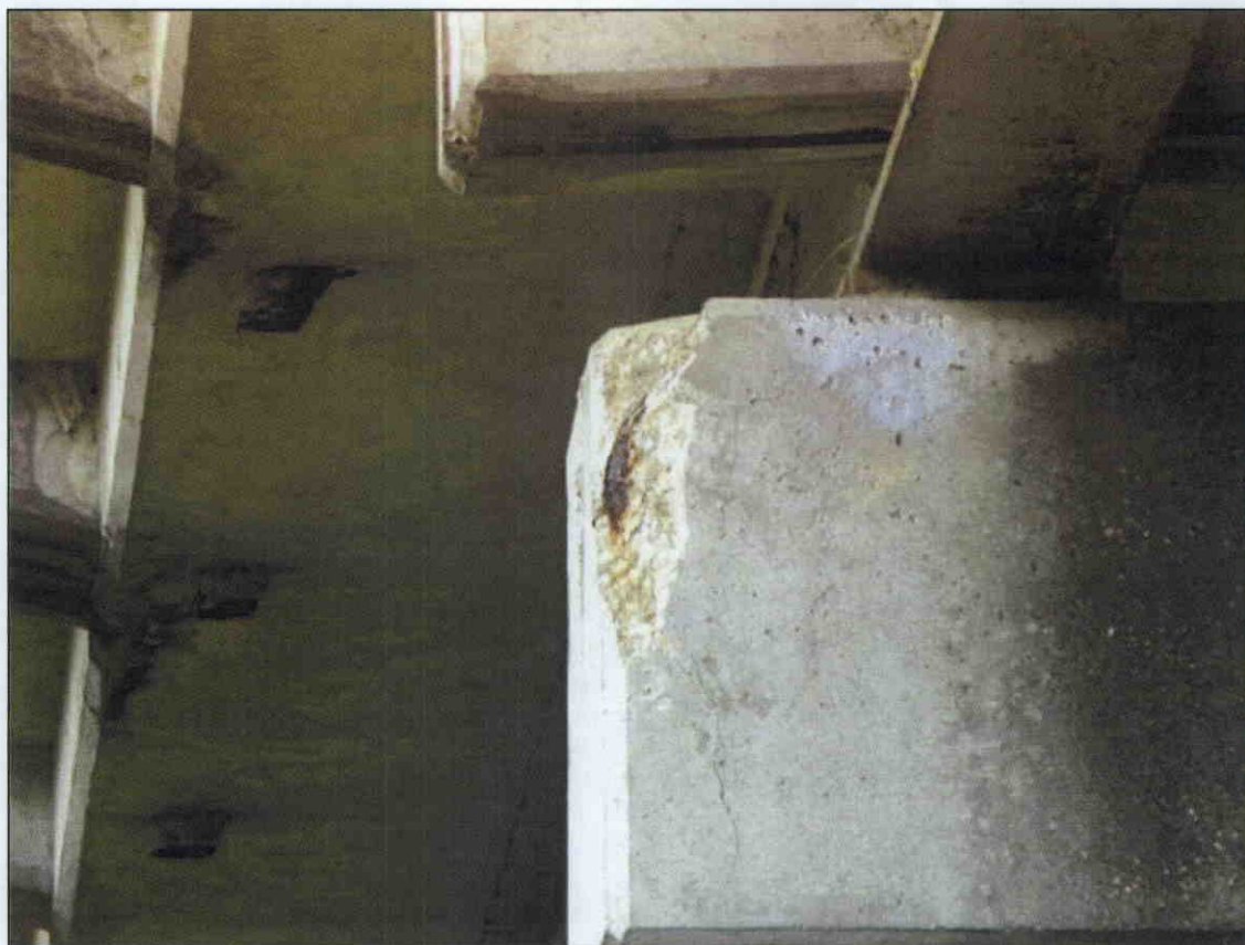
CORNER SPALL WITH EXPOSED REBAR AT BENT 1 RIGHT END OF CAP
