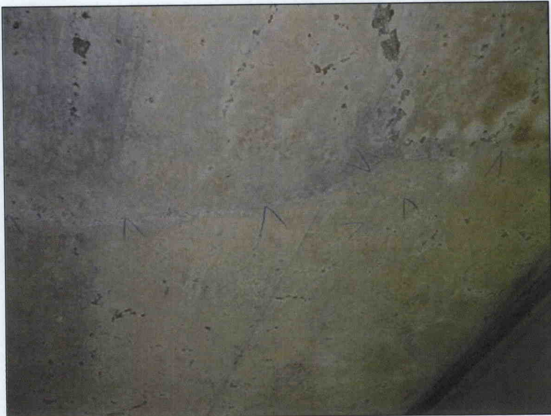
HAIRLINE MAP CRACKING IN BOTTOM OF DECK SPAN 1
