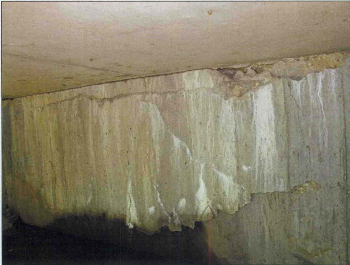
BACKWALL AT END BENT 2 BAY 2 CRACKED, SPALLED AND DELAMINATING
