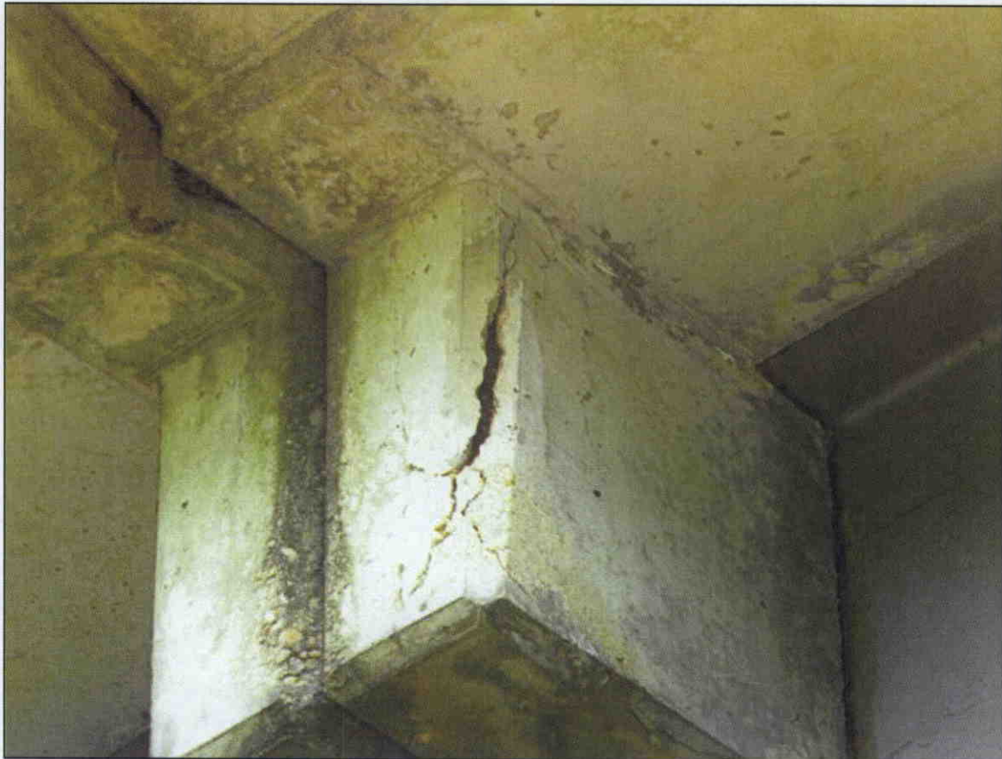
LEFT EXTERIOR DIAPHRAGM AT BENT 3 SPAN 3 SIDE CRACKED AND DELAMINATING
