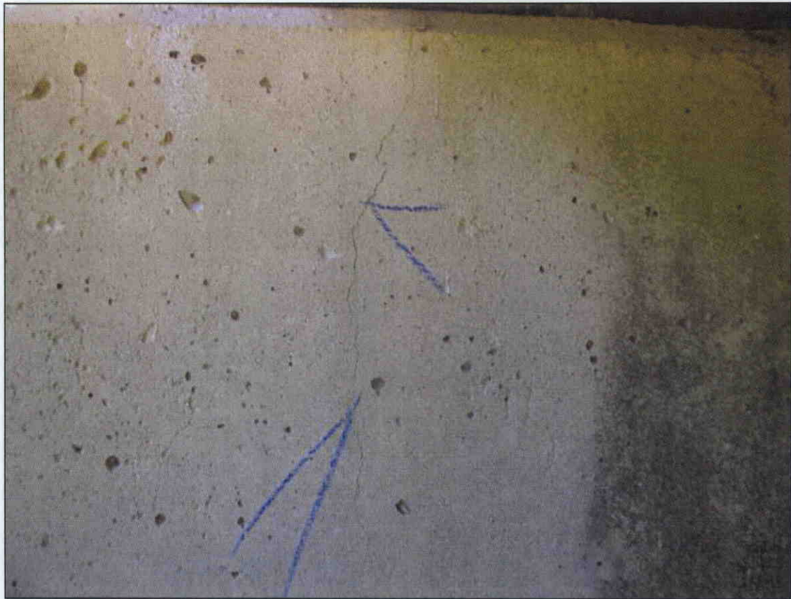
HAIRLINE VERTICAL CRACK IN FACE OF CAP AT BENT 2 SPAN 3 SIDE UNDER BEAM 4
