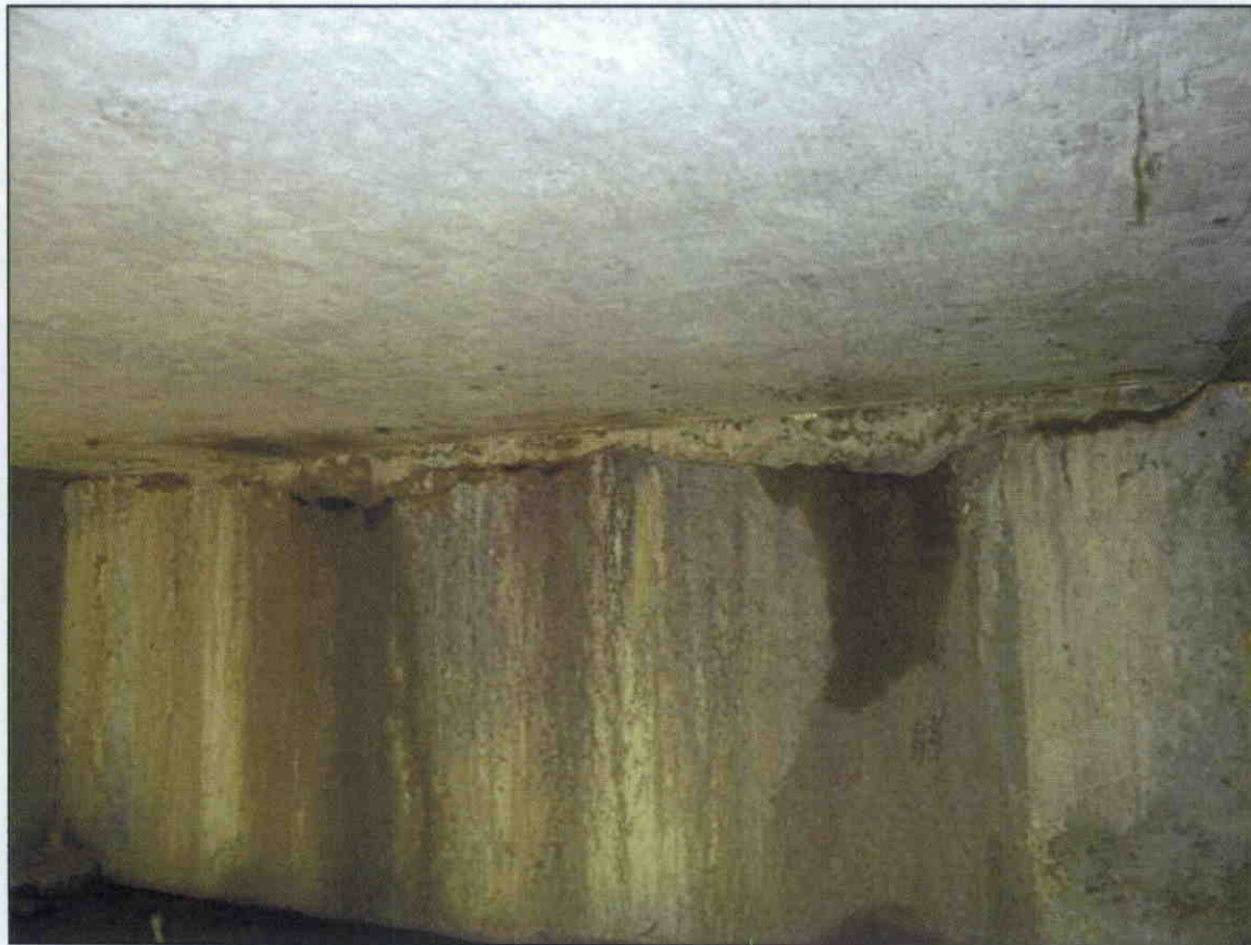
DELAMINATION ALONG THE TOP OF BACKWALL AT END BENT 2 BAY 1
