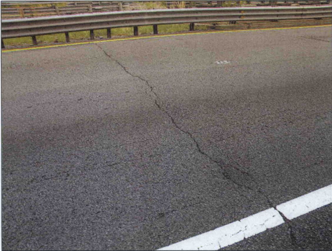
TRANSVERSE CRACK IN APPROACH 2
