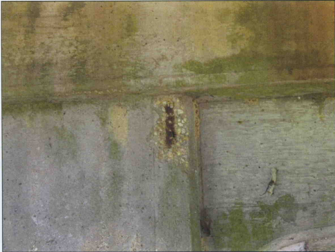
SURFACE SPALL WITH EXPOSED REBAR IN COLUMN 1 AT BENT 1 SPAN 1 SIDE JUST UNDER CAP
