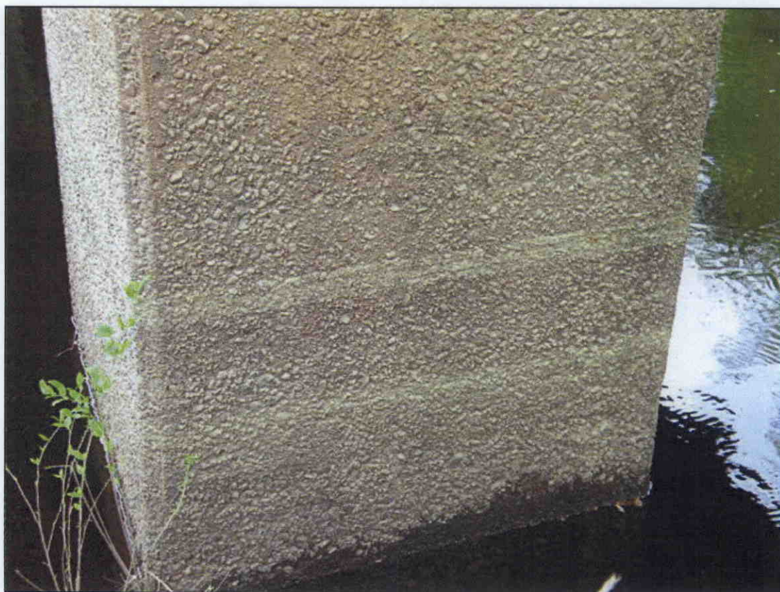
BENT COLUMNS SCALED WITH COARSE AGGREGATE EXPOSED UP TO HIGH WATER MARK
