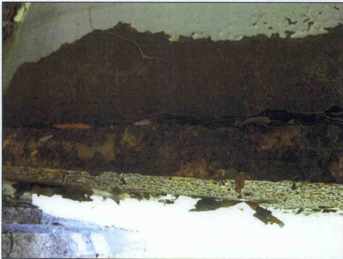
SECTION LOSS IN THE RIGHT SIDE BOTTOM FLANGE AND WEB OF BEAM 1 IN SPAN 3 OVER BENT 2
