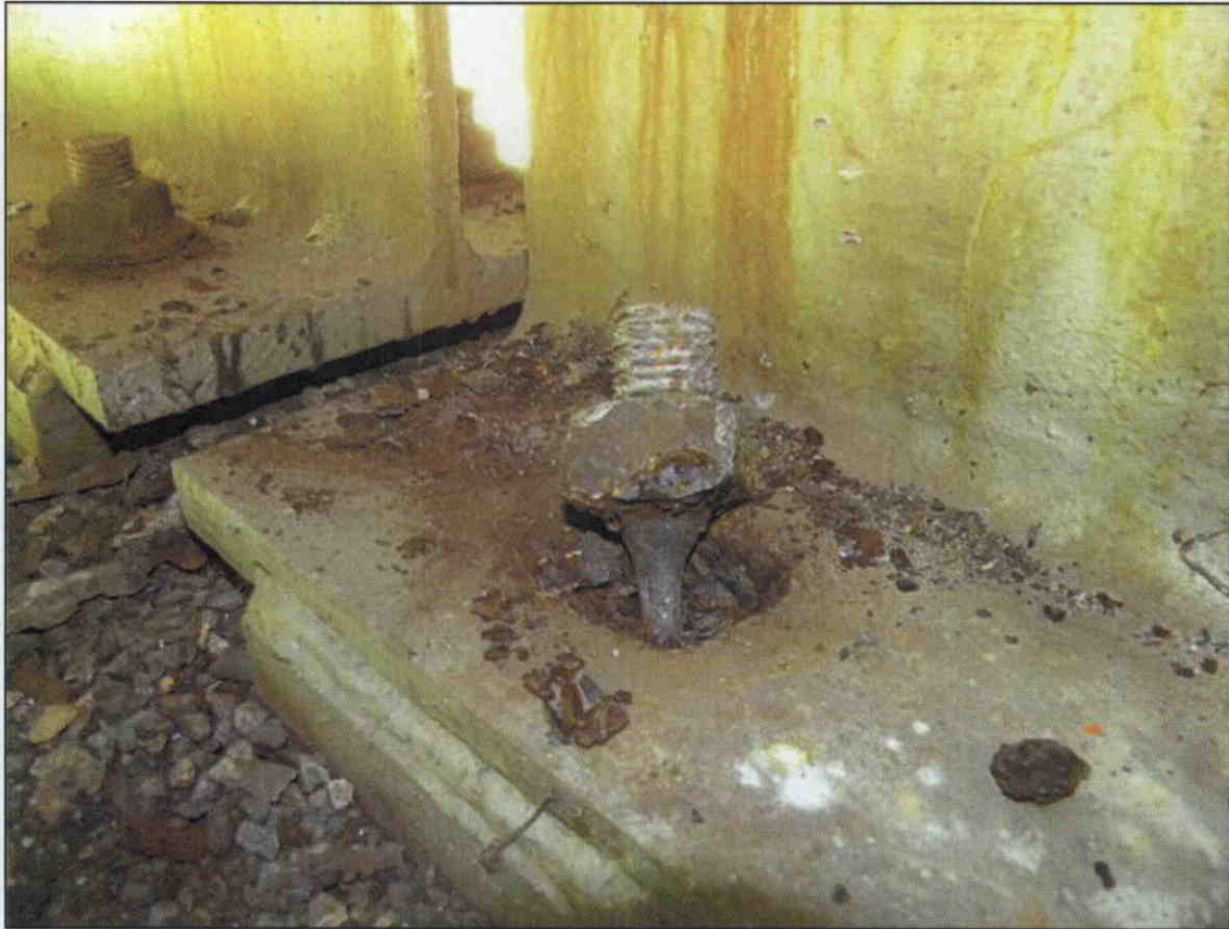
SECTION LOSS IN THE LEFT SIDE ANCHOR BOLT OF BEAM 2 BEARING ASSEMBLY AT BENT 3 SPAN 3 SIDE (PRIORTIY MAINTENACE ISSUED)
