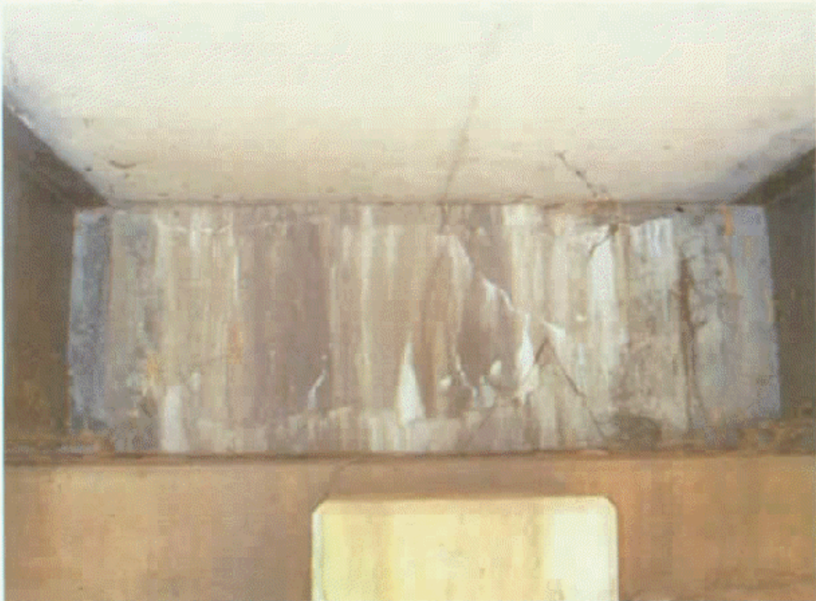
BAY 2 AT END BENT 2 CURTAINWALL CRACKING W/ EFFLO.
