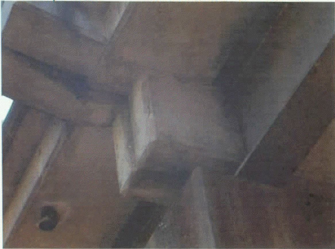
SPAN 3 AT BENT 3 W. END DIAPH. SPALLED & DELAM.
