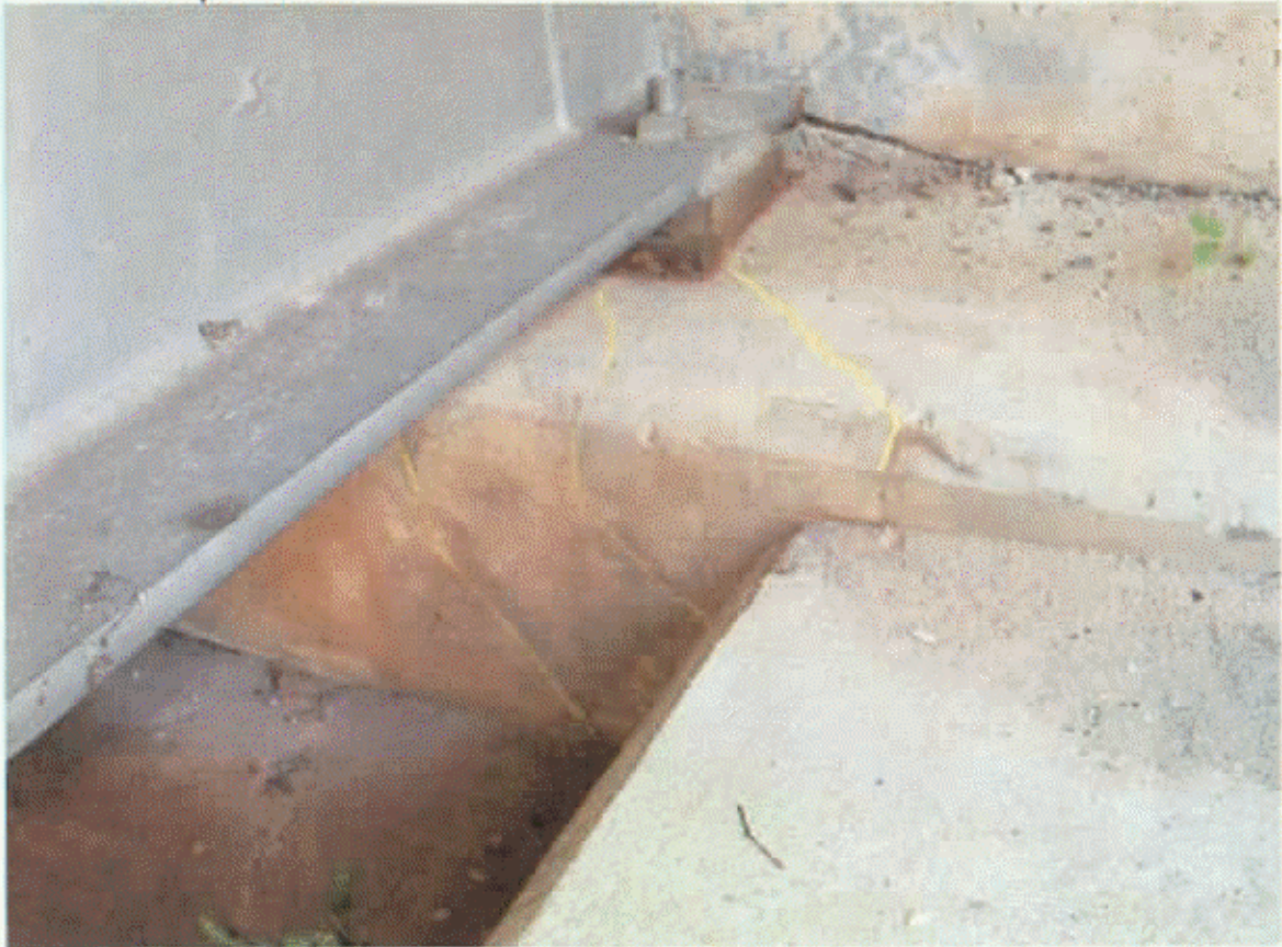
END BENT 1 CAP AT BRACE PILE NO. 1 DIAGONAL CRACKS
