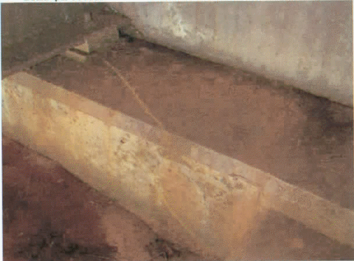
END BENT 1 CAP AT BRACE PILE 2 CRACKED AT BEAM 3
