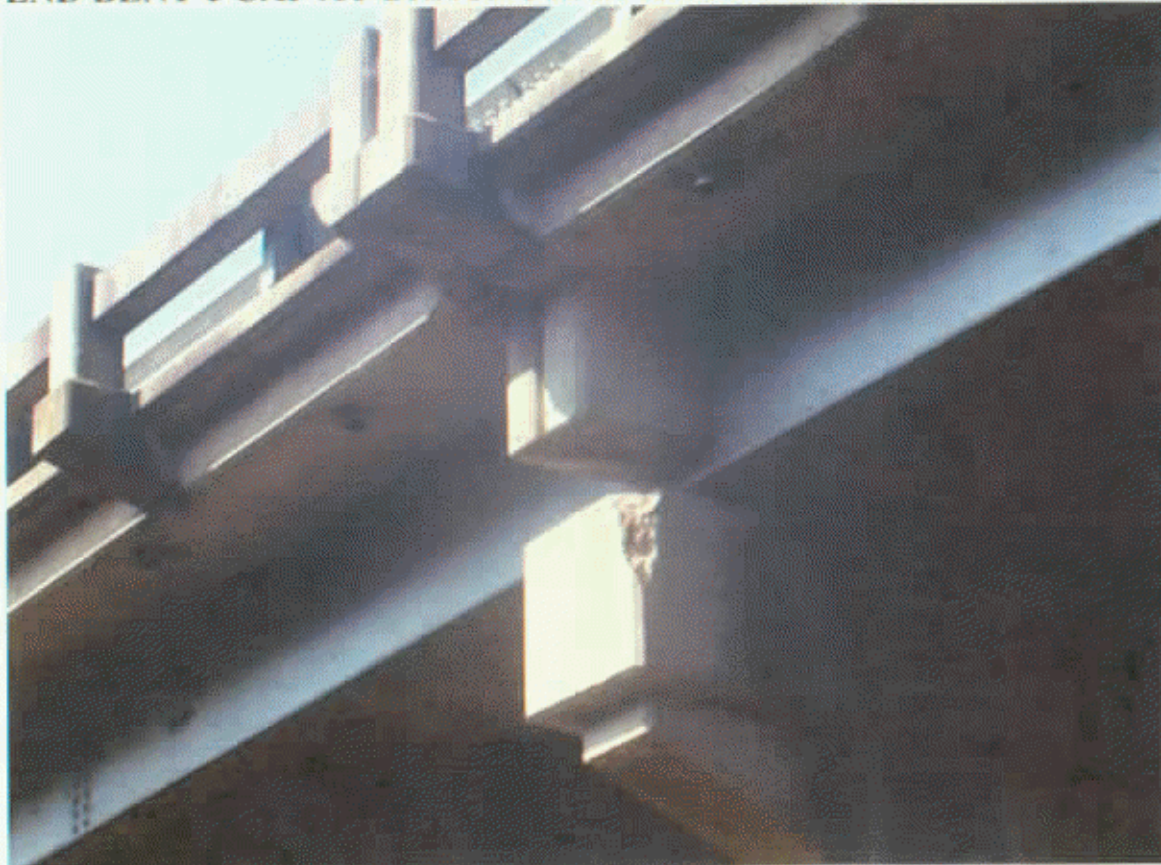
BENT 1 CAP @ EAST END SPALLED & SPAN 1 RAIL SPALLED
