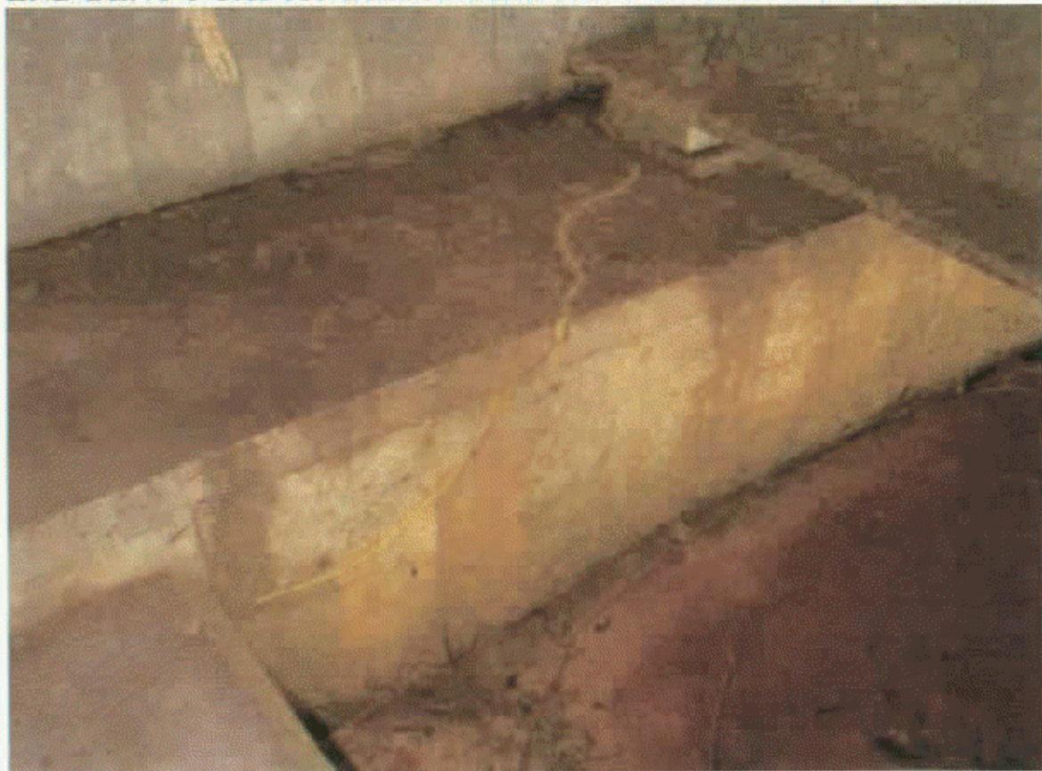
END BENT 1 CAP @ BRACE PILE NO. 2 CRACKED
