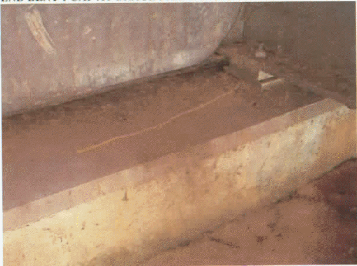
END BENT 1 CAP AT BAY 3 CRACKED TO BEAM 3
