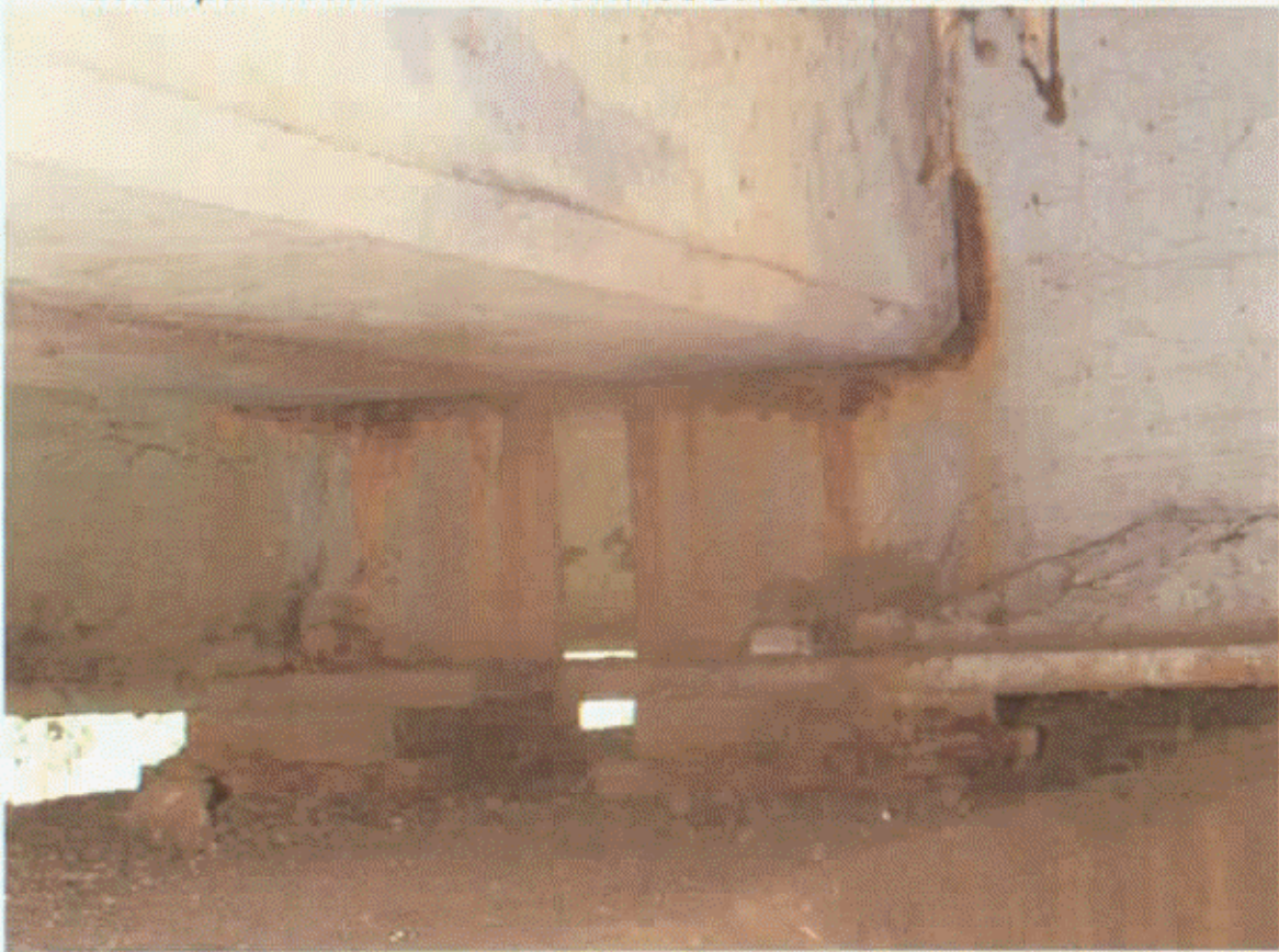
BEAM 3 IN SPANS 1, AND 2 AT BENT 1 BEAM RUST
