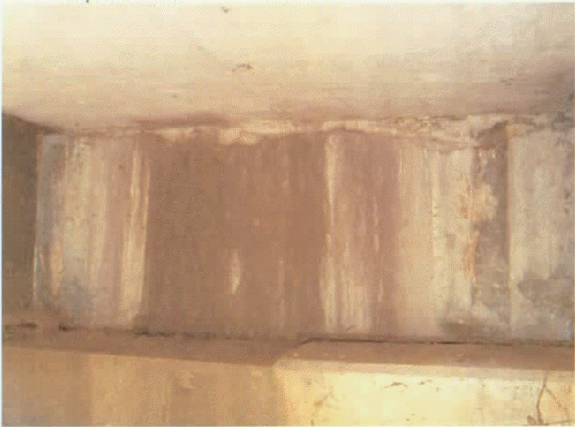
BAY 1, END BENT 2 CURTAINWALL CRACK & LEAKAGE
