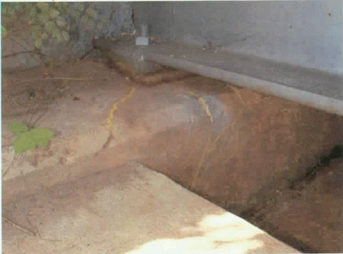
END BENT 1 CAP AT BRACE PILE NO. 3 CRACKING
