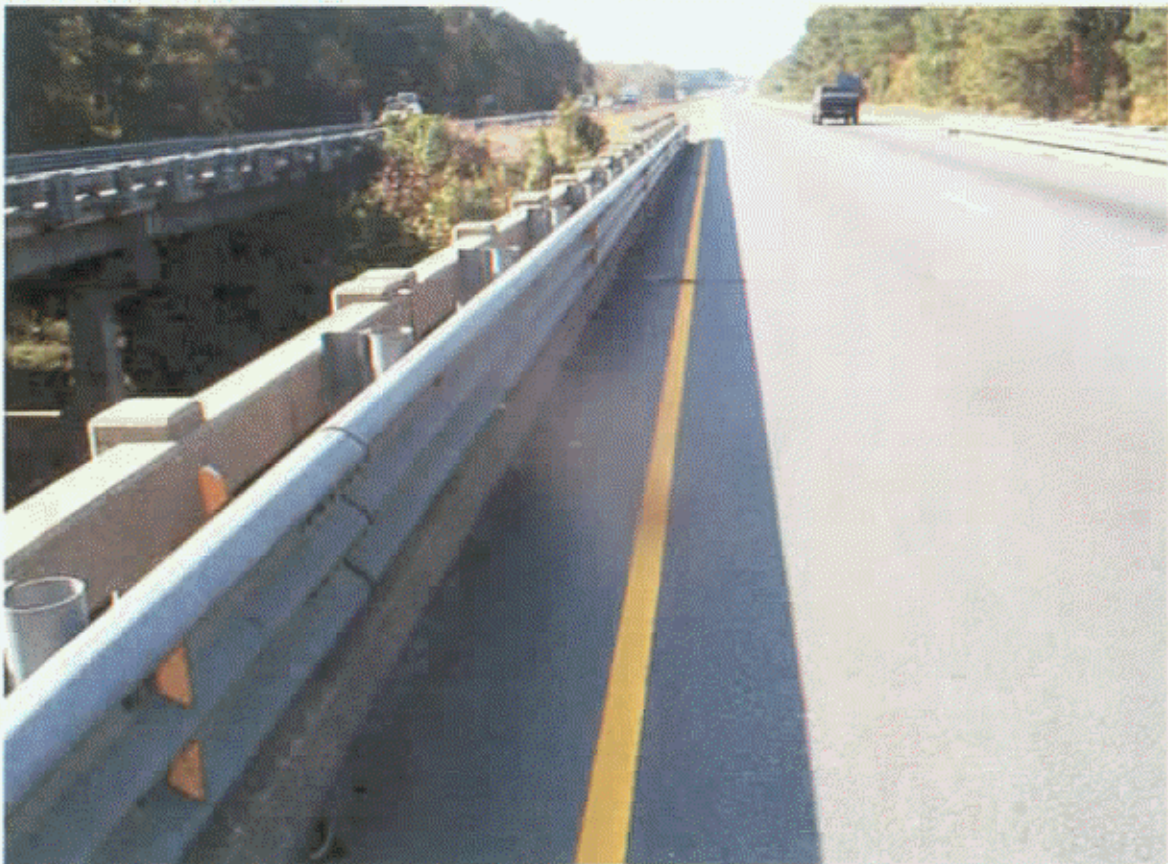
DEBRIS ALONG THE EAST RAIL.
