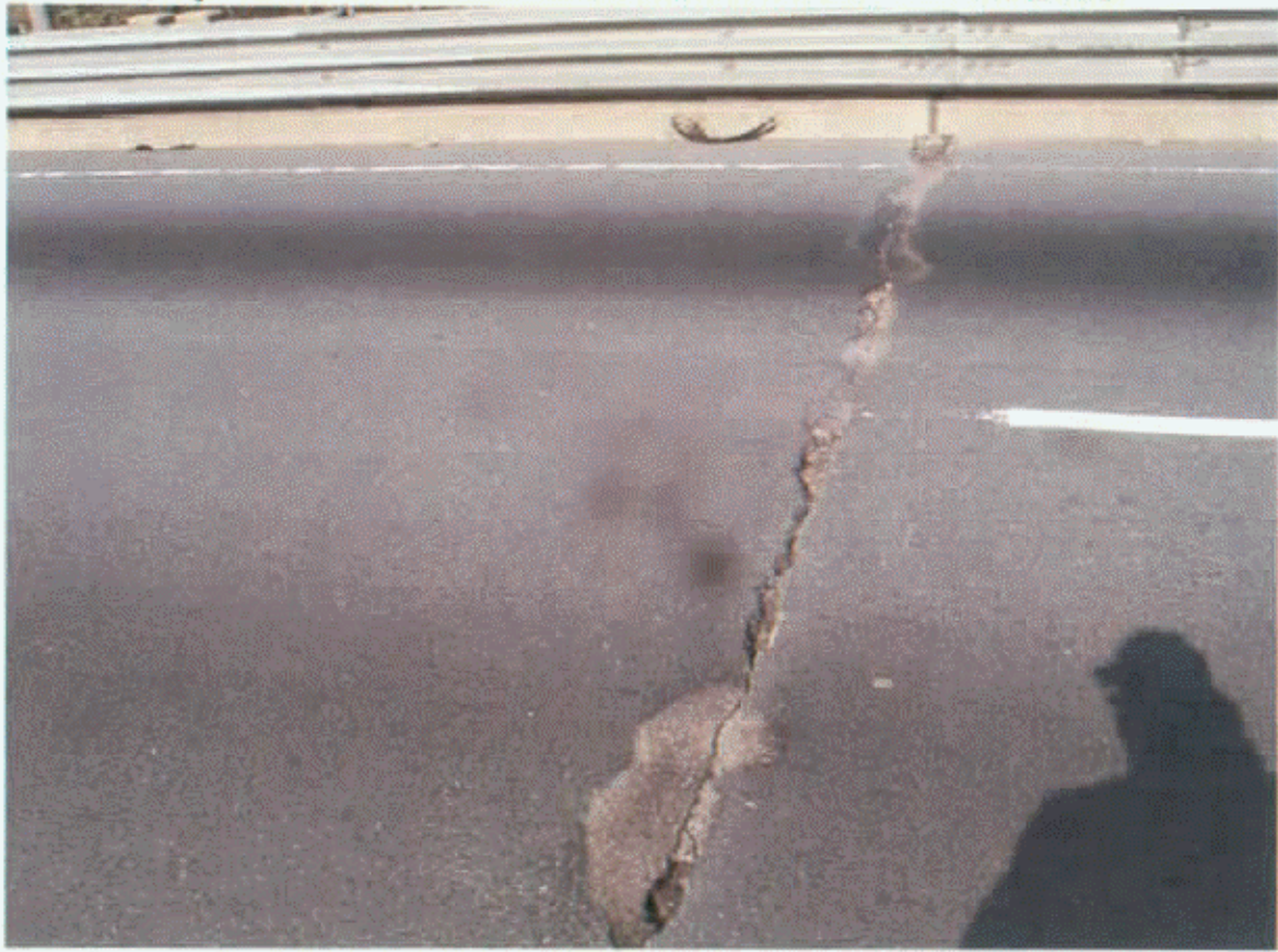
ASPHALT WEARING SURFACE AT BENT 3 JOINT
