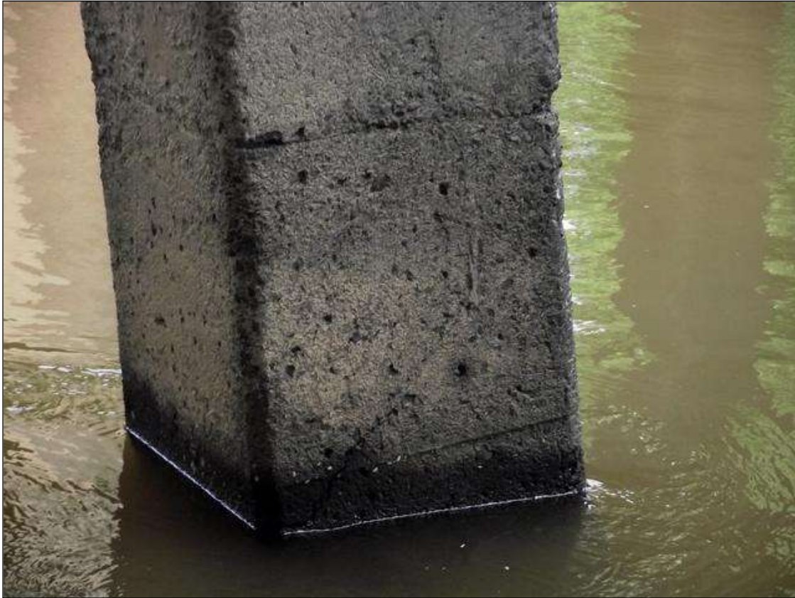
PILES IN WATERWAY HAVE WATER ABRASION WITH THE EXPOSED AGGREGATE IN FLOWZONE.
