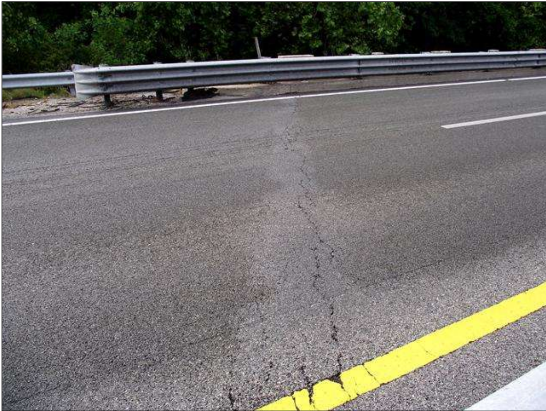
TRANSVERSE CRACKING IN WEARING SURFACE OVER END BENT 2
