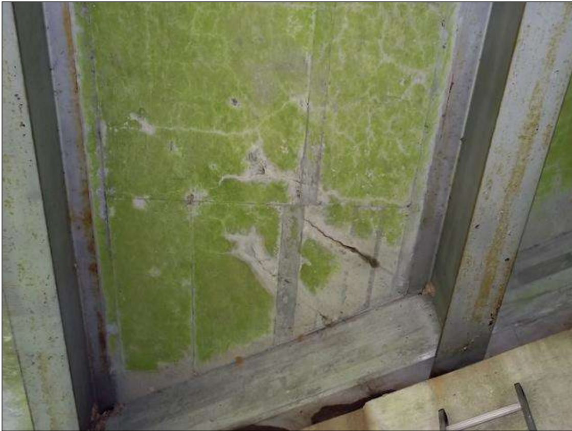
HAIRLINE DIAGONAL CRACKS IN BOTTOM OF DECK OF SPAN 2 BAY 1 AT BENT 2
