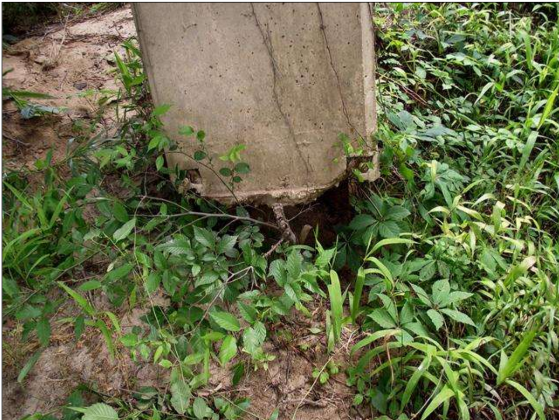
BOTTOM OF PILE 7 CONCRETE ENCASEMENT UNDERMINED WITH SECTION LOSS TO EXPOSED STEEL H-PILE
