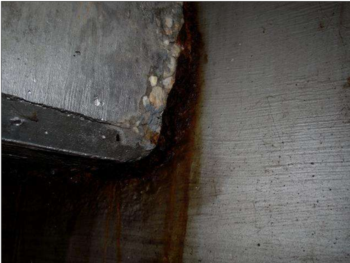
SECTION LOSS IN THE WEB OF BEAM 3 AT JUNCTION OF DIAPHRAGM SPAN 1 OVER BENT 1
