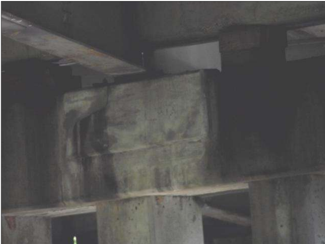
SPALL REPAIR IN FACE OF CAP AT BENT 4 BAY 3 SPAN 4 SIDE
