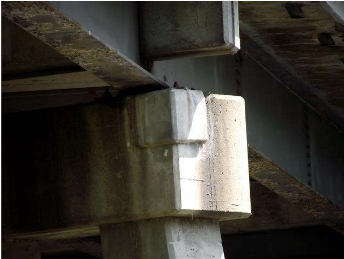
SPALL REPAIR IN RIGHT END OF CAP AT BENT 4
