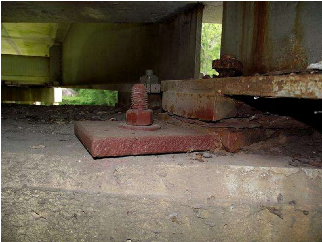
ANCHOR BOLT REPAIR AT BEAM 4 OVER BENT 2 - OTHER REPAIRS SIMILAR AT THIS BENT
