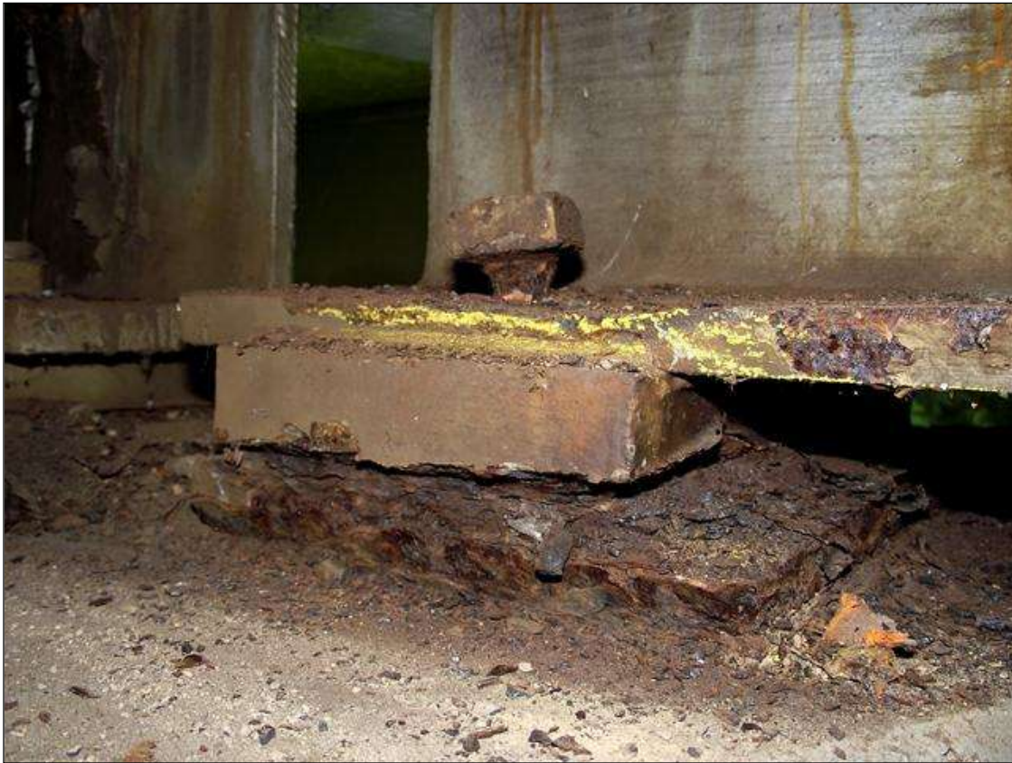
SECTION LOSS IN THE BOTTOM FLANGE OF BEAM 3 IN SPAN 1 OVER BENT 1
