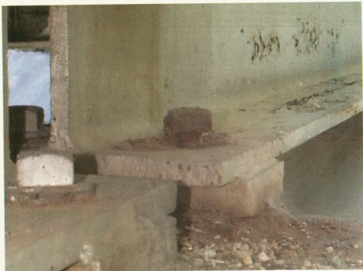
BT 6, SP 6, BM 4, RT ANCHOR BOLT HEAVILY RUSTED AND PUSHED UP
