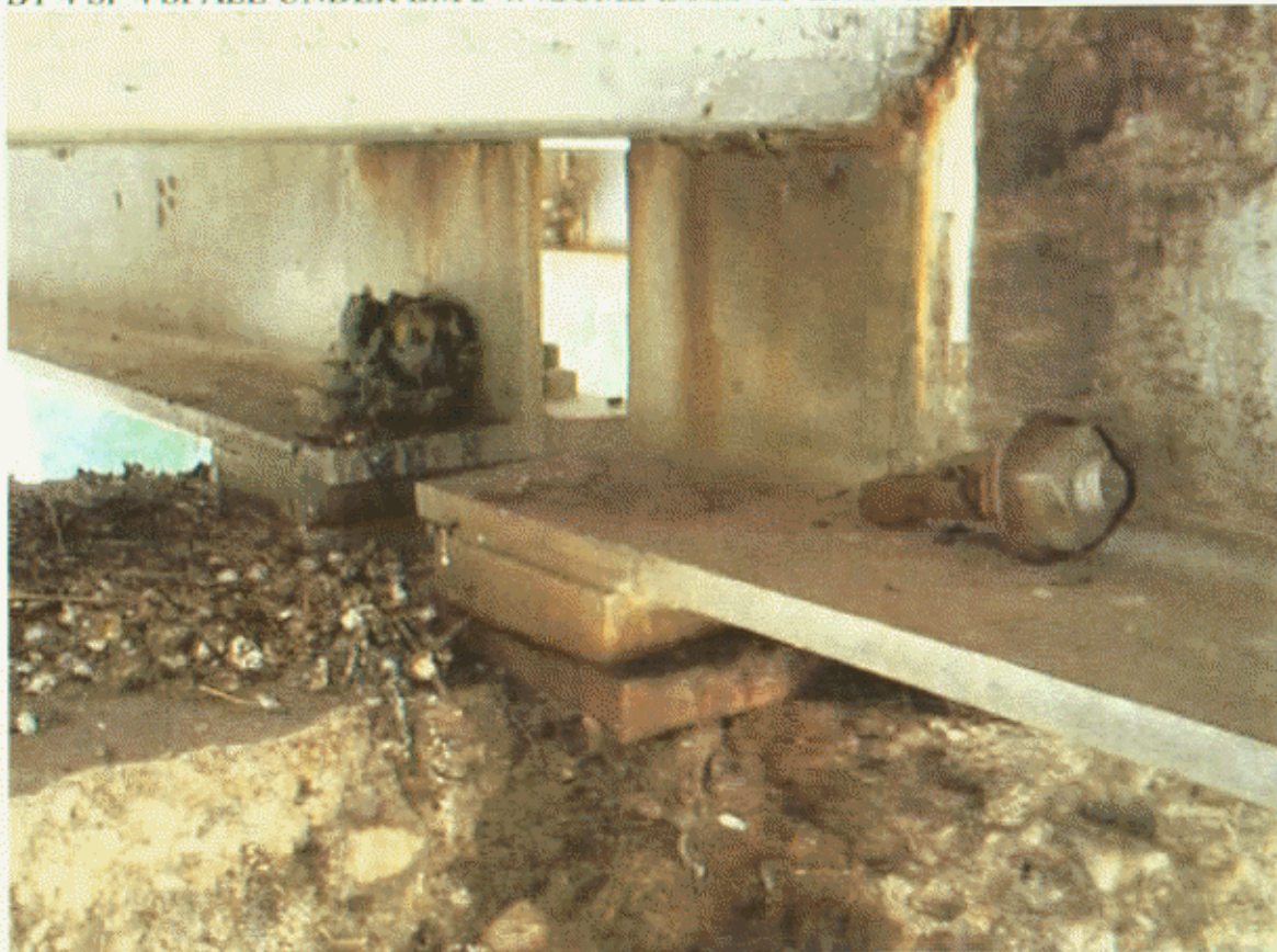
BT 4 SP 4, LT ANCHOR BOLT AT BM 3 IS BROKEN OFF
