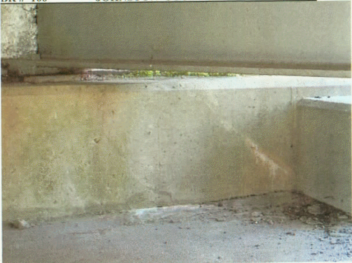
EB 1, BAY 2 CAP HAS DIAG H/L CR AT BRACE PILE CAP 1 AND BM 1 HAS RUSTING BRG
