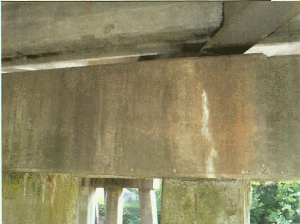
BT 3 SP 3 VERT H/L CR IN CAP AT P-5 FROM TOP TO BOTTOM
