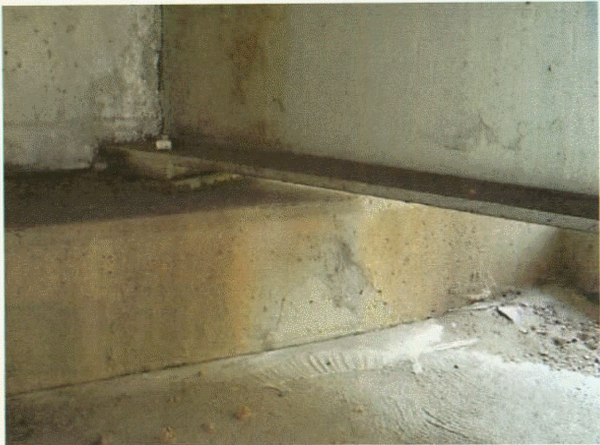
EB 2 AT BM 4, H/L TO 1/32" CRS IN FACE AND TOP OF CAP, SIMILAR AT BM
