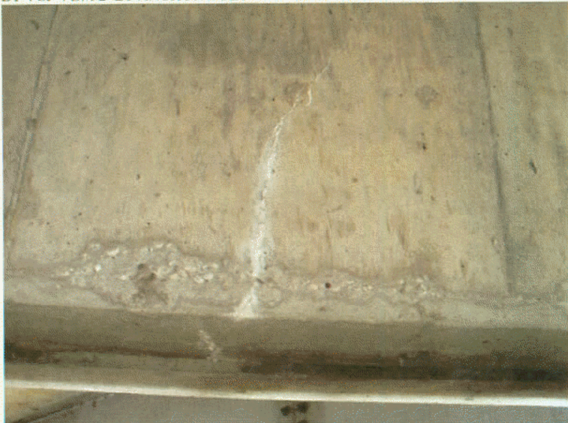
BT 4 SP 4 BAY 1 DIAPH CR DOWN FACE AND ACROSS BOTTOM.
