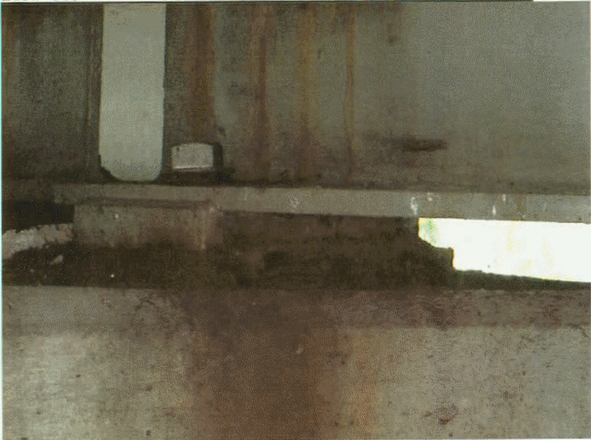
BT 6 , SP7 , RT ANCHOR BOLT AND BRG. HEAVILY RUSTED
