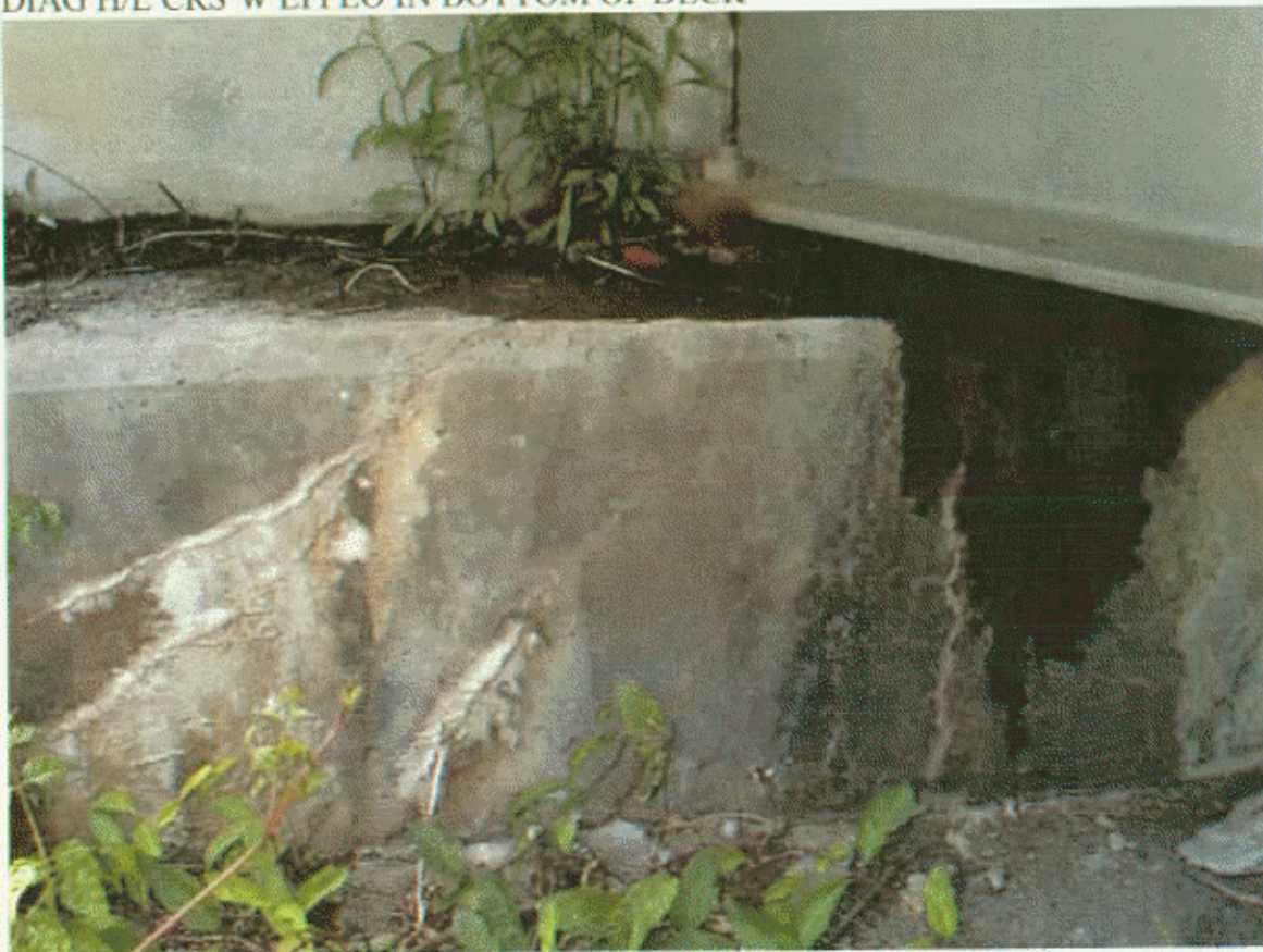
EB 1 AT BM 4 , BRG IS RUSTED AND FLAKING ALSO WATER STANDING ON CAP AND CAP IS H/L CR INFACE AND ON TOP
