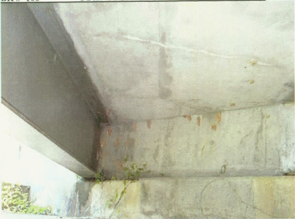
AT E B 1 , BAY 3 , CAP HAS VERT AND DIAG H/L CRS SOME W EFFLO AND DIAG H/L CRS W EFFLO IN BOTTOM OF DECK
