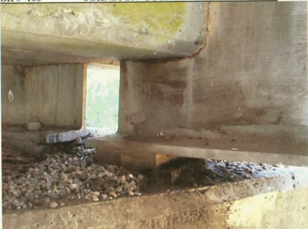
BT 4 SP 4 ,BM4, LT ANCHOR BOLT RUSTED INTO
