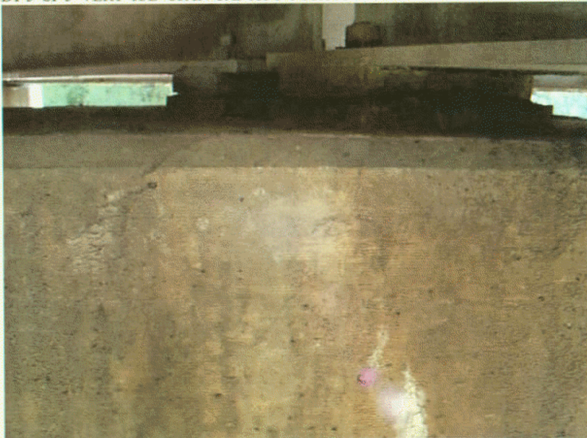
BT 3 SP 3 BM3 , CRS IN TOP ND FACE , RUNNING BACK TO ANCHOR BOLTS
