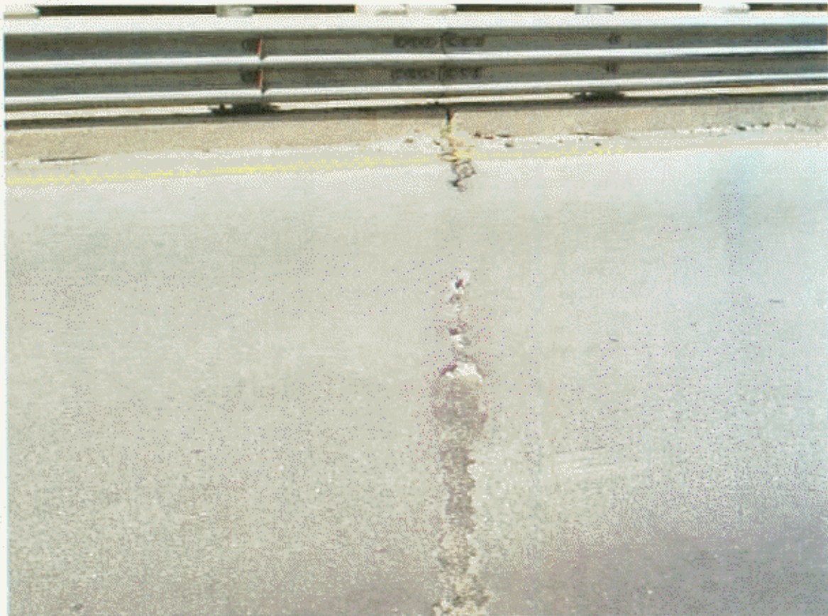
EXP JT AT BT 7- A W S CR OR MISSING AND , SIMILAR AT ALL JOINTS
