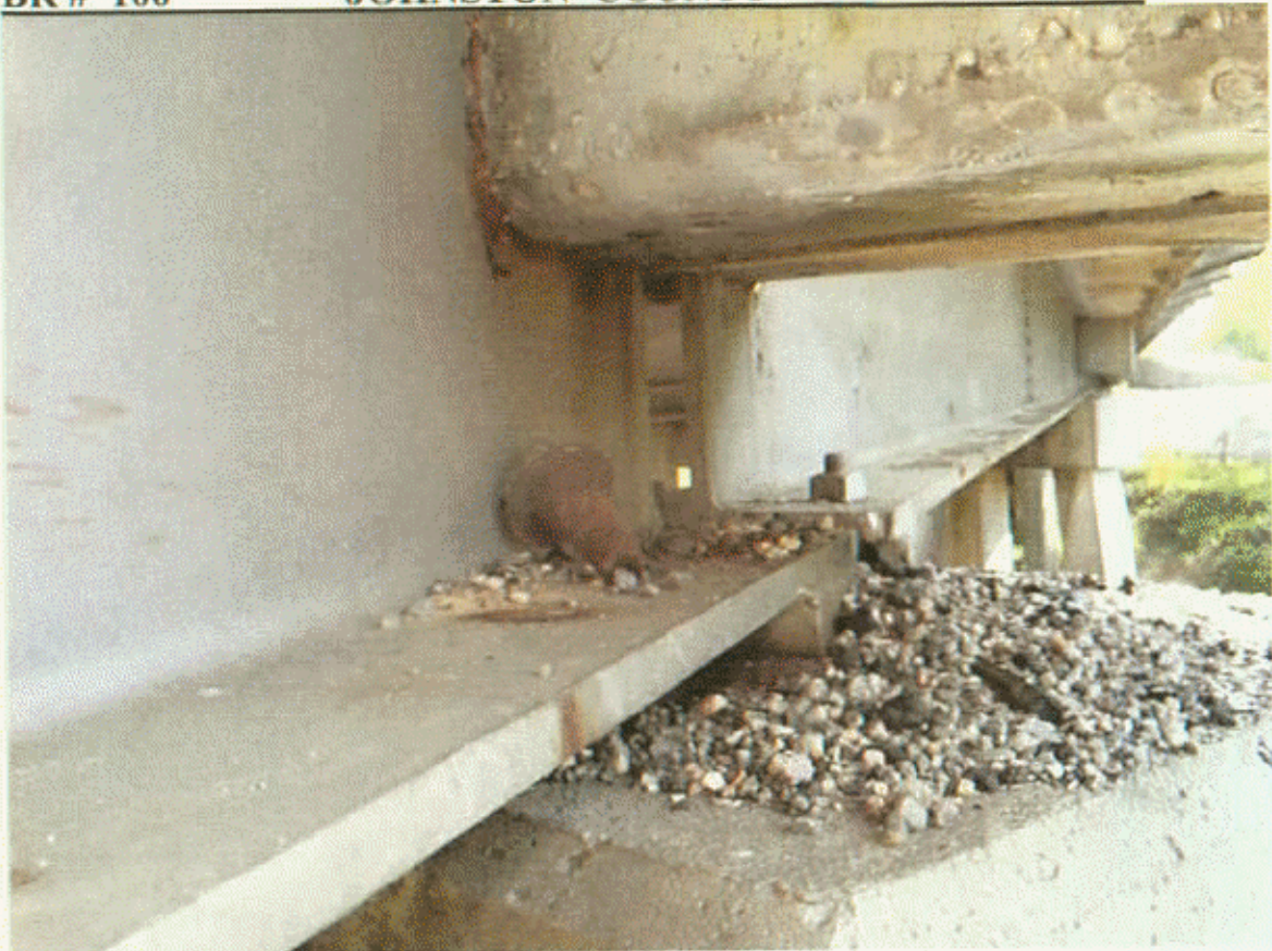
BT 4 SP 4, BM 4 RT ANCHOR BOLT BROKEN OFF
