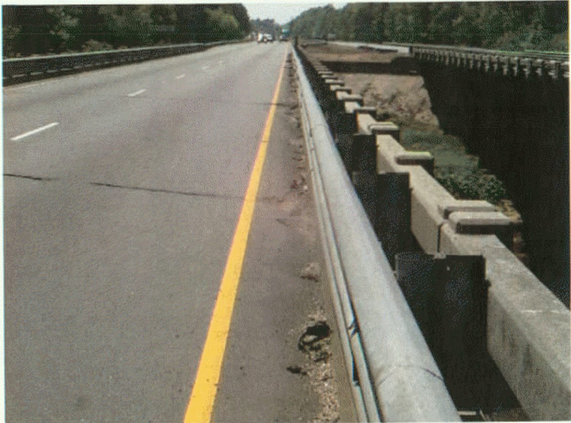
DEBRIS AT LT CURB, SIMILAR AT RT.
