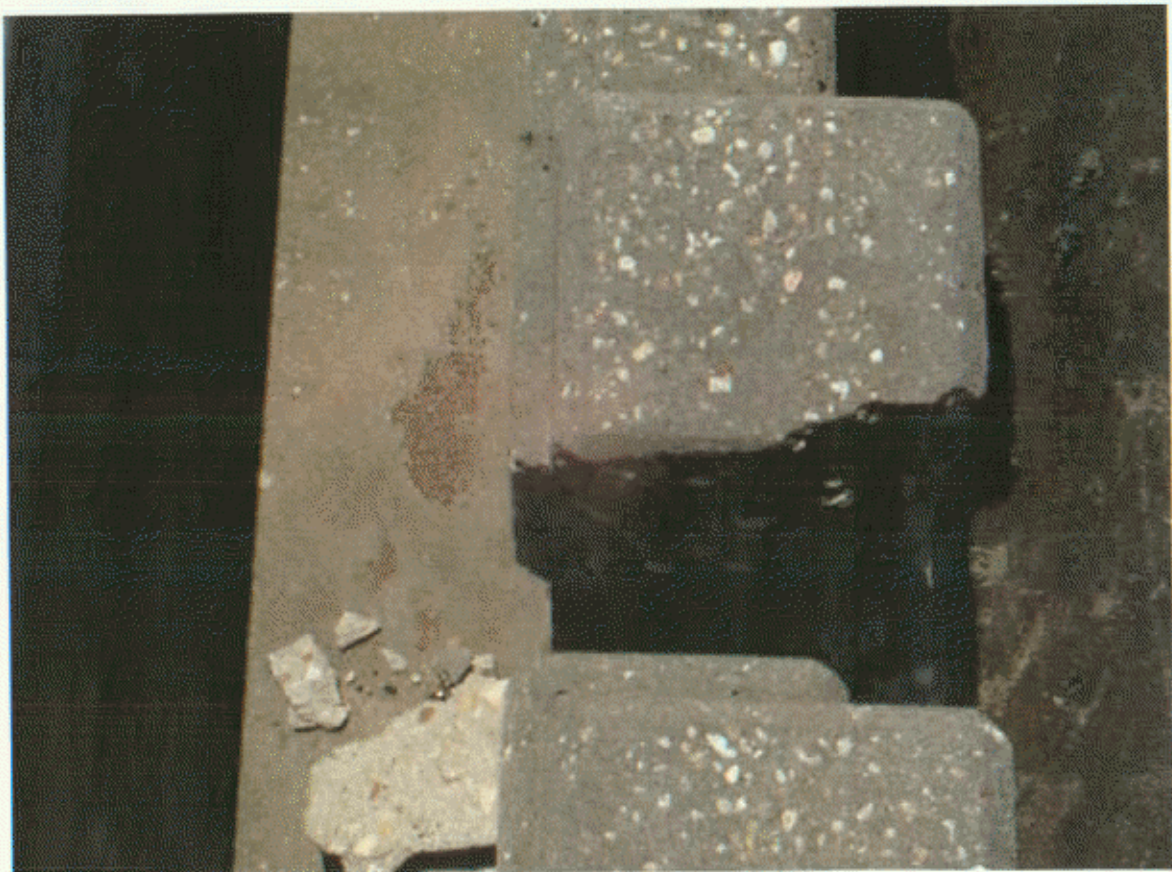
SP 1, LT RAIL POST #3 SPALLED
