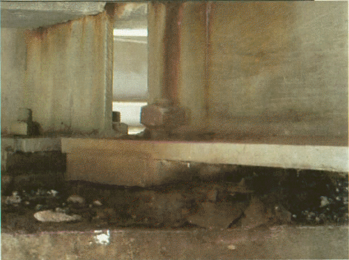
BT 4 SP 4 BM 2 LT ANCHOR BOLT AND BRG HEAVILY RUSTED
