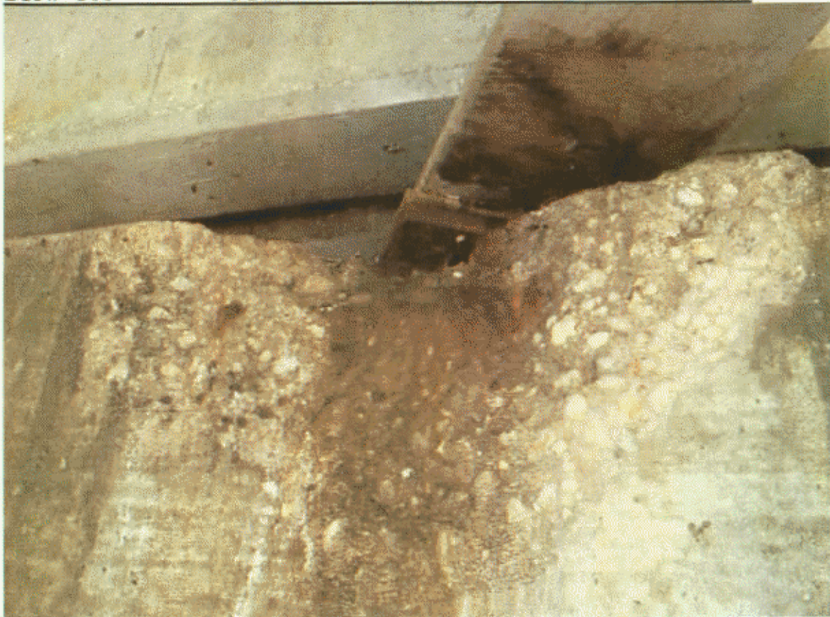
BT 4 SP 4 SPALL UNDER BM 3 W /SOME LOSS OF BRG AREA
