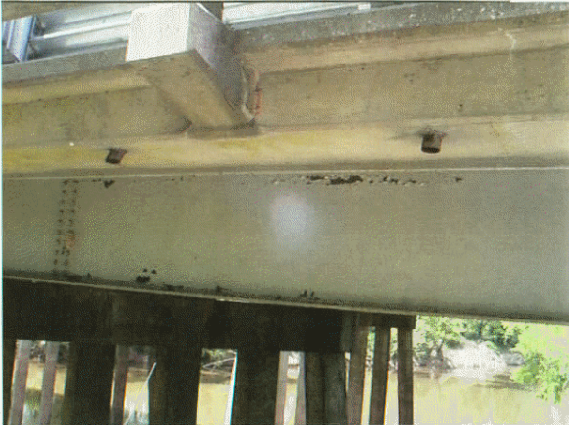
SP 8, BM 4, PAINT PEELING , FEW OTHERS SIMILAR IN ALL SPANS
