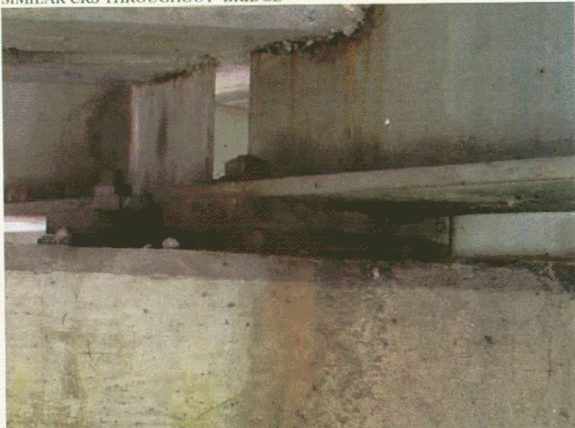
BT 2 SP 2 BM 2 BRG RUSTING ,NUMEROUS OTHERS SIMILAR THROUGHOUT BRIDGE
