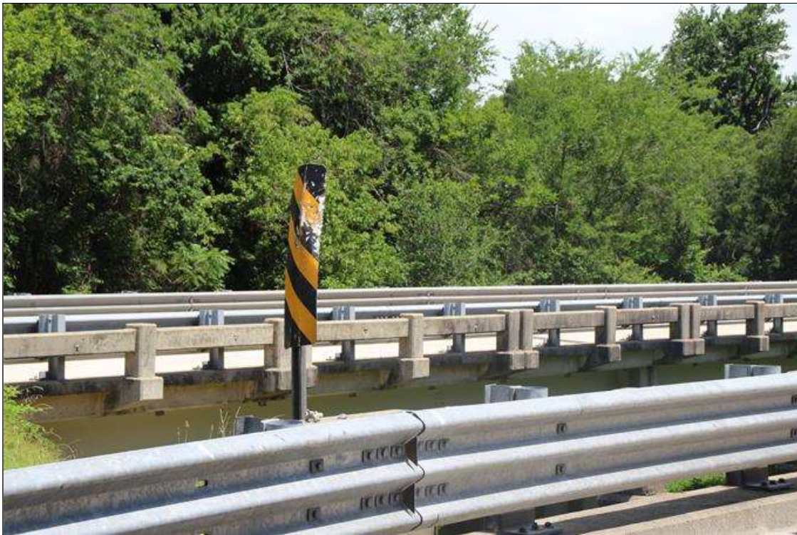
MODERATE IMPACT DAMAGE TO DELINEATOR AT SOUTHWEST CORNER.
