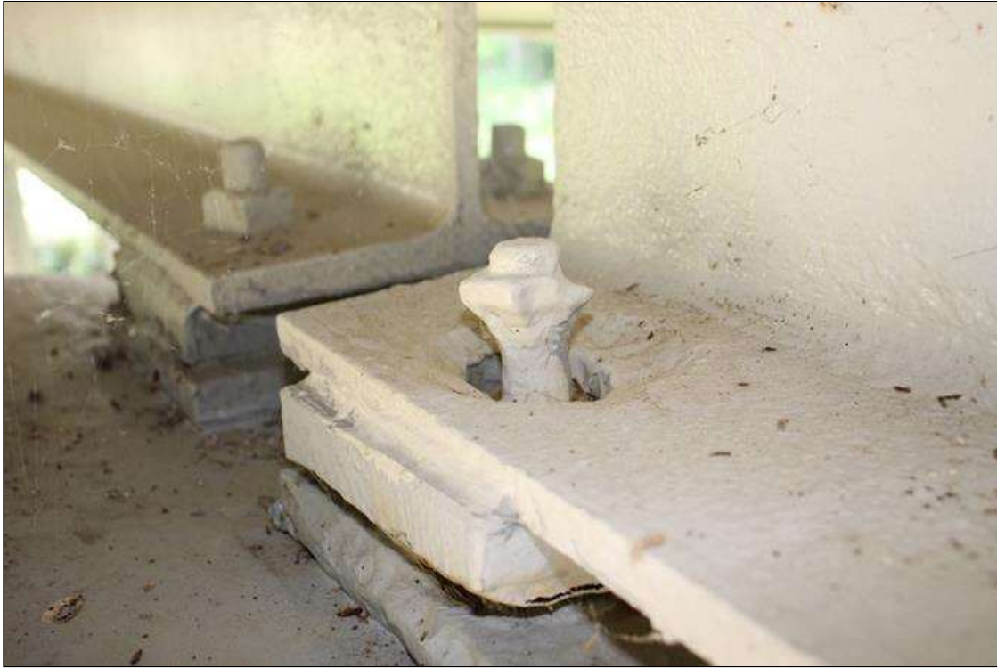
Span 6 Beam 3 Far Bearing: LEFT ANCHOR BOLT HAS UP TO 80% SECTION REMAINING AND ANCHOR BOLT NUT HAS UP TO 50% SECTION REMAINING.
