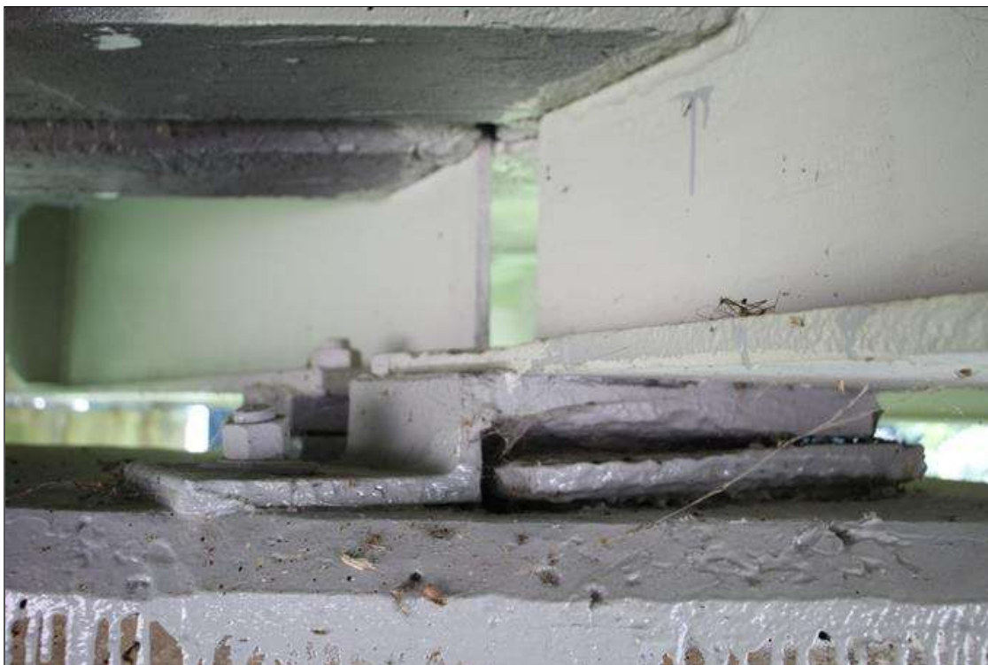
PREVIOUS REPAIR TO FAR BEARING IN SPAN 1 BEAM 3. TYPICAL AT BEAM 1.
