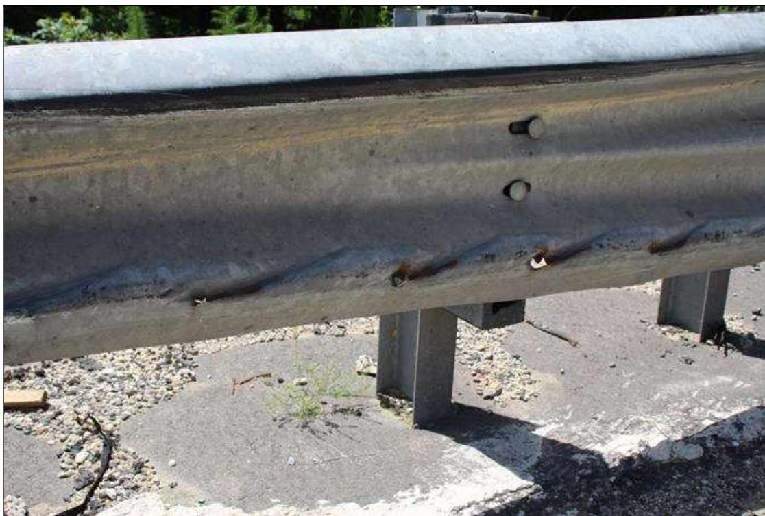
HEAVY IMPACT DAMAGE WITH UP TO 1.5 IN DIAMETER HOLES IN THE APPROACH GUARDRAIL TRANSITION AT NORTHEAST CORNER. FOR 25 FT LONG STARTING AT END BENT 1
