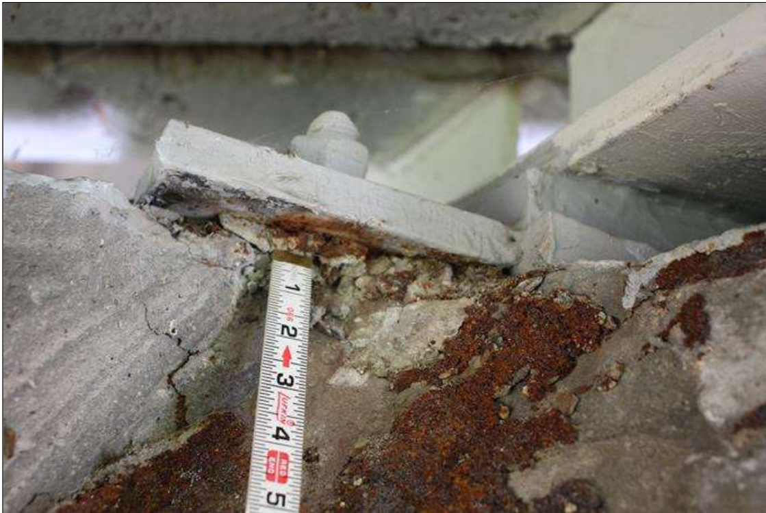
Span 4 Beam 3 Far Bearing: NEW BEARING HAS A LOSS OF BEARING AREA DUE TO SPALL ON CAP. 5 IN WIDE X 1 IN DEEP AREA OF BEARING PLATE IS UNDERMINED (PAR).
