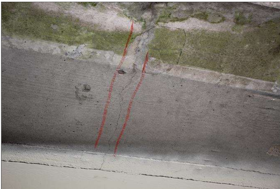
Span 1 Deck: SIX (6) UP TO 0.02 IN WIDE TRANSVERSE CRACKS UNDER LEFT OVERHANG, SCATTERED.
