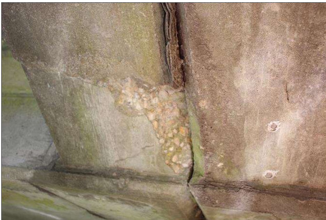
Span 1 Deck: 9 IN LONG X UP TO 4 IN WIDE X UP TO 2.5 IN DEEP SPALL IN RIGHT DECK OVERHANG ABOVE BENT 1.
