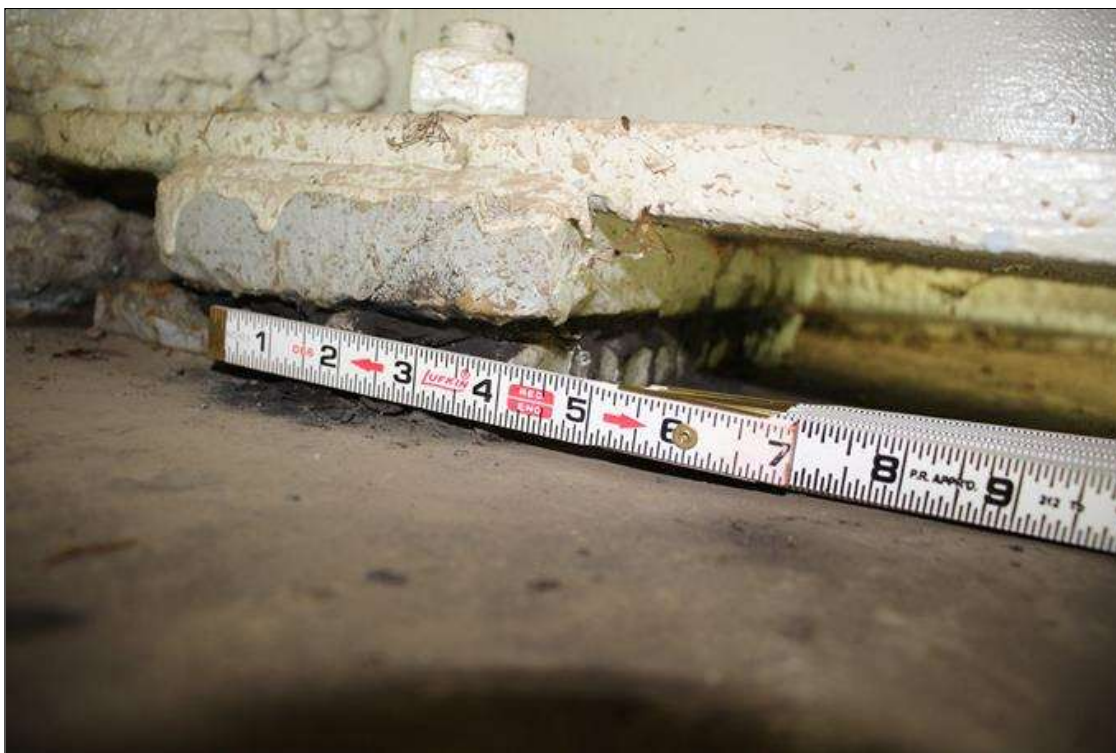
Span 8 Beam 4 Far Bearing: UP TO 1/2 IN MOVEMENT TOWARDS THE SOUTH LEFT HALF OF THE MASONRY PLATE.
