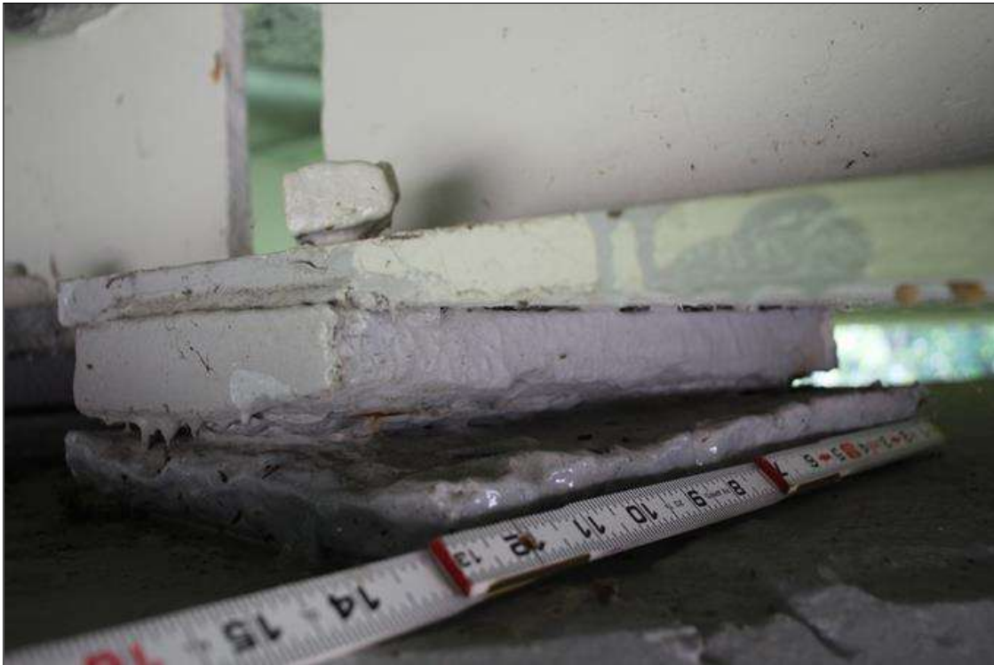
Span 1 Beam 2 Far Bearing: BEARINGS HAVE BEEN PAINTED SINCE PREVIOUS INSPECTION. SECTION LOSS EXISTS BENEATH THE PAINTED SURFACES IN BOTH MASONRY AND SOLE PLATES. UP TO 80% SECTION REMAINING.
