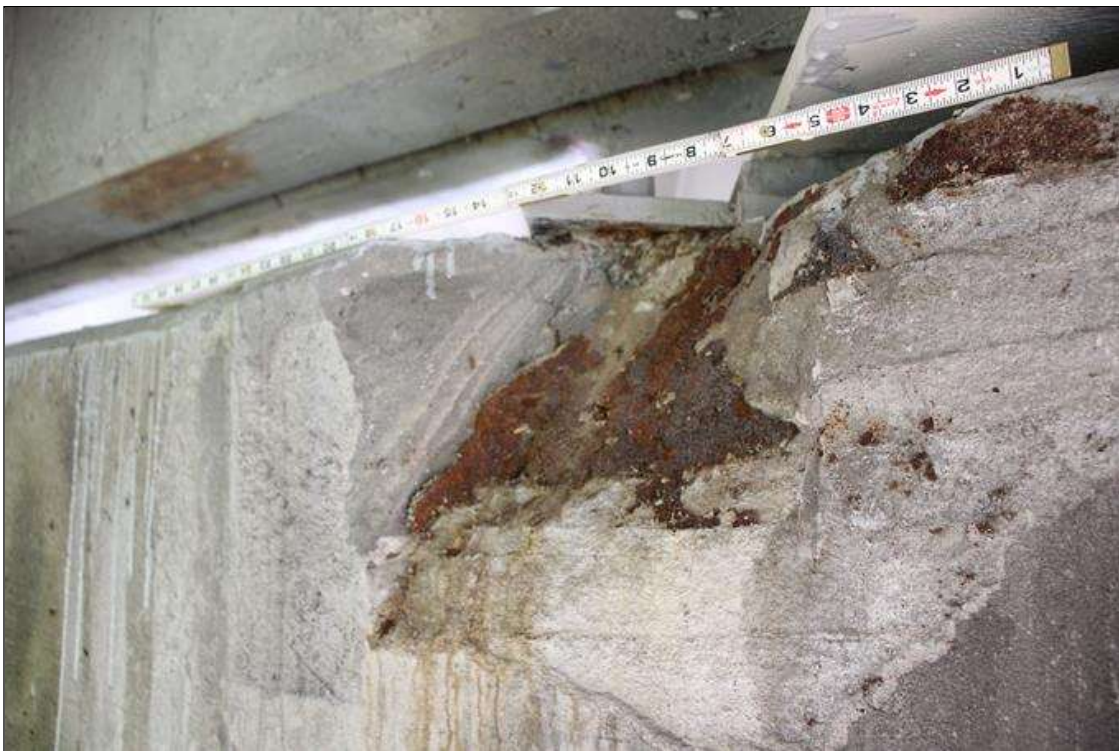
Bent 4 Cap 1: 17 IN WIDE X UP TO 11 IN HIGH X UP TO 6 IN DEEP SPALLED PATCHED AREA, TOP OF SOUTH FACE, EXTENDING BELOW BEAM 3 BEARING ASSEMBLY, BEARING IS NOT SEATED LEVEL (PAR).
