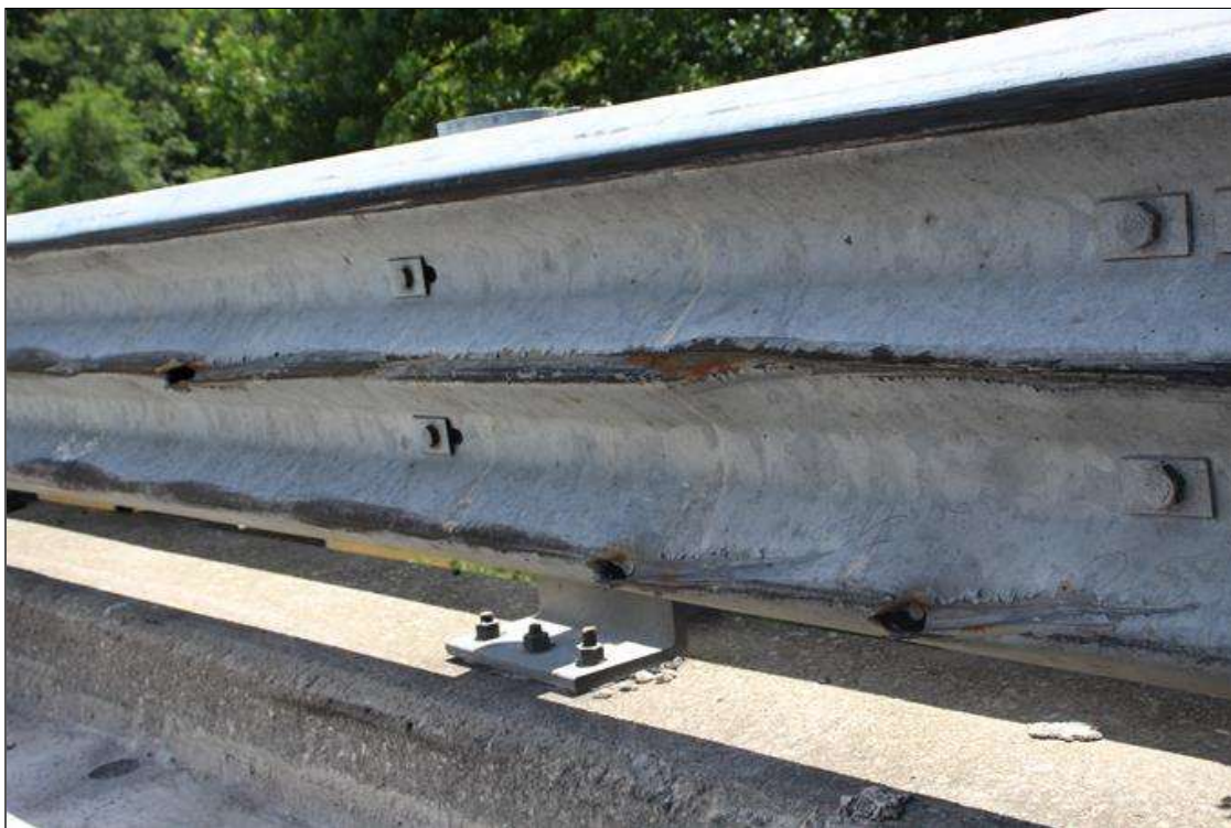
HEAVY IMPACT DAMAGE WITH 1 IN WIDE CRACK AND 4 IN WIDE X 1 IN HIGH HOLES IN RIGHT BRIDGE RAIL AT END BENT 1.
