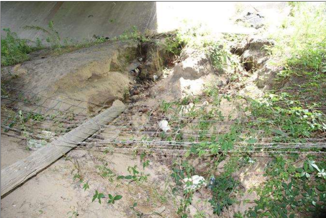
9 FT WIDE X 15 FT LONG X UP TO 3 FT DEEP AREA OF EROSION UNDER SPAN 8 WITH BROKEN AND FALLEN FENCE POSTS.
