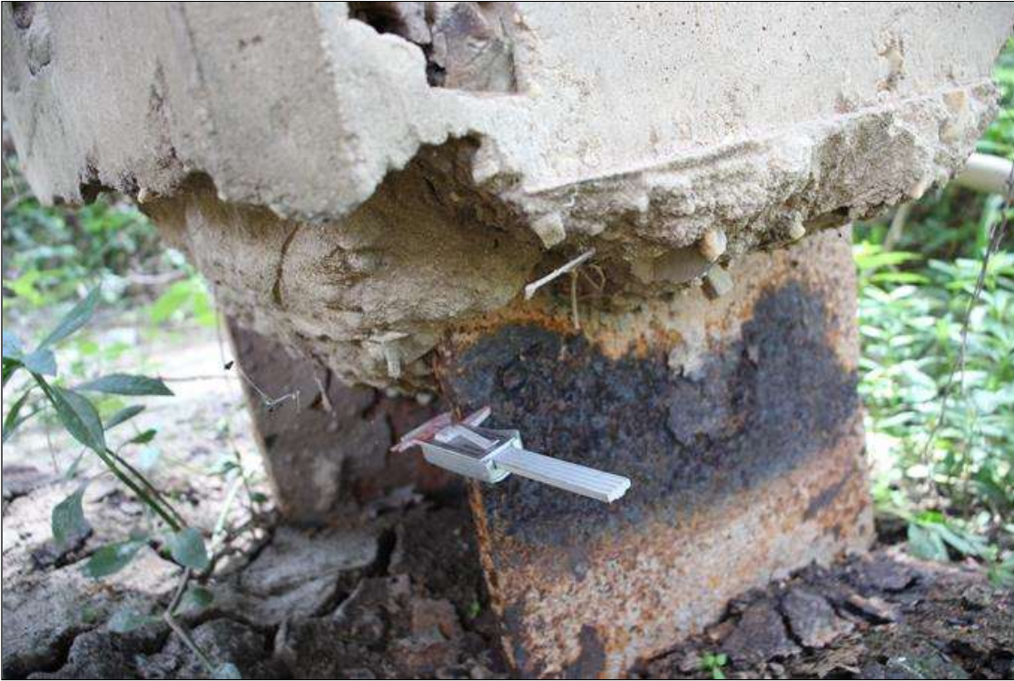
Bent 7 Pile 7: 15 IN WIDE X 10 IN HIGH AREA OF THE SOUTH FLANGE EXHIBITS HEAVY SURFACE CORROSION WITH SECTION LOSS ON WEB AND FLANGES OF EXPOSED STEEL PILE AT GROUNDLINE. UP TO 0.50 IN SECTION REMAINING (PAR). NORTH FLANGE AND THE WEB EXHIBIT HEAVY SURFACE CORROSION WITH NO MEASUREABLE SECTION LOSS.
