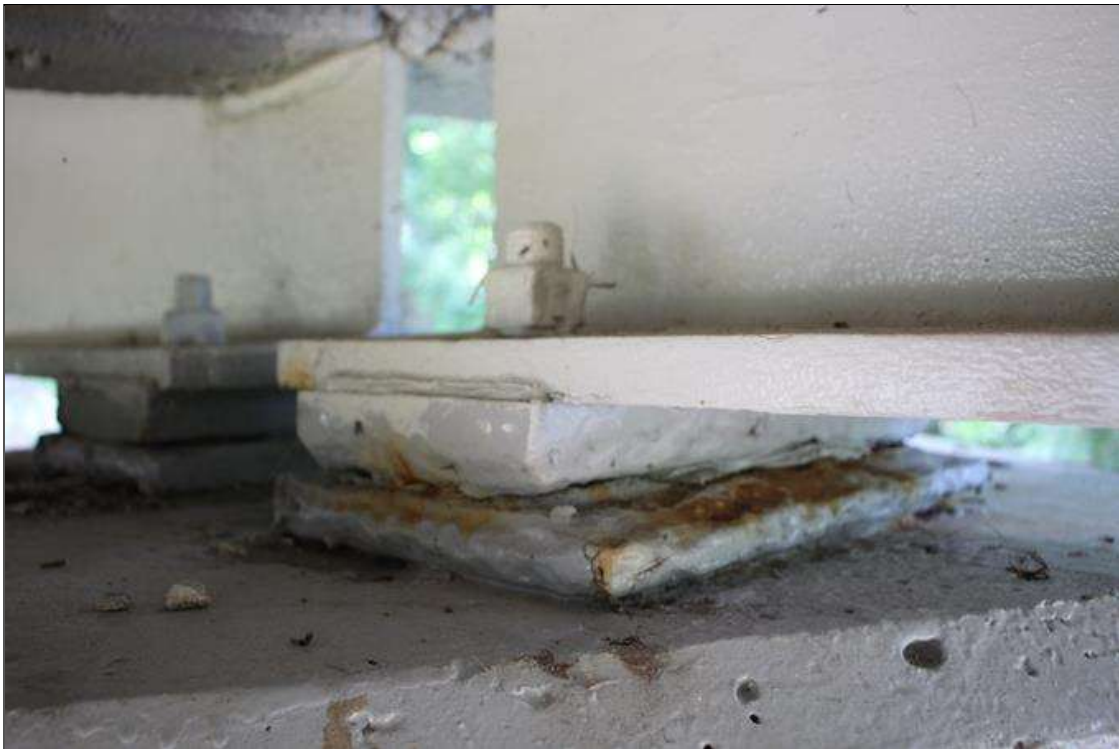
Span 6 Beam 4 Far Bearing: BEARINGS HAVE BEEN PAINTED SINCE PREVIOUS INSPECTION. SECTION LOSS EXISTS BENEATH THE PAINTED SURFACES IN BOTH MASONRY AND SOLE PLATES. UP TO 80% SECTION REMAINING. RUST STAINING PRESENT IN NEWLY PAINTED SURFACES.
