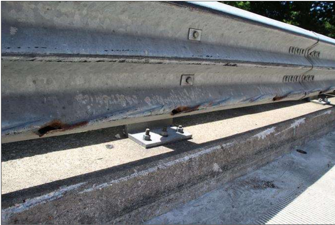
Span 8 Right Bridge Rail: HEAVY IMPACT DAMAGE WITH UP TO 3 IN LONG X 1 IN HIGH HOLES AND DENTS IN THE BOTTOM OF CONCRETE SUPPLMENTAL BRIDGE RAIL FOR FULL SPAN LENGTH. DAMAGE EXTENDS INTO SPANS 7 AND 6.
