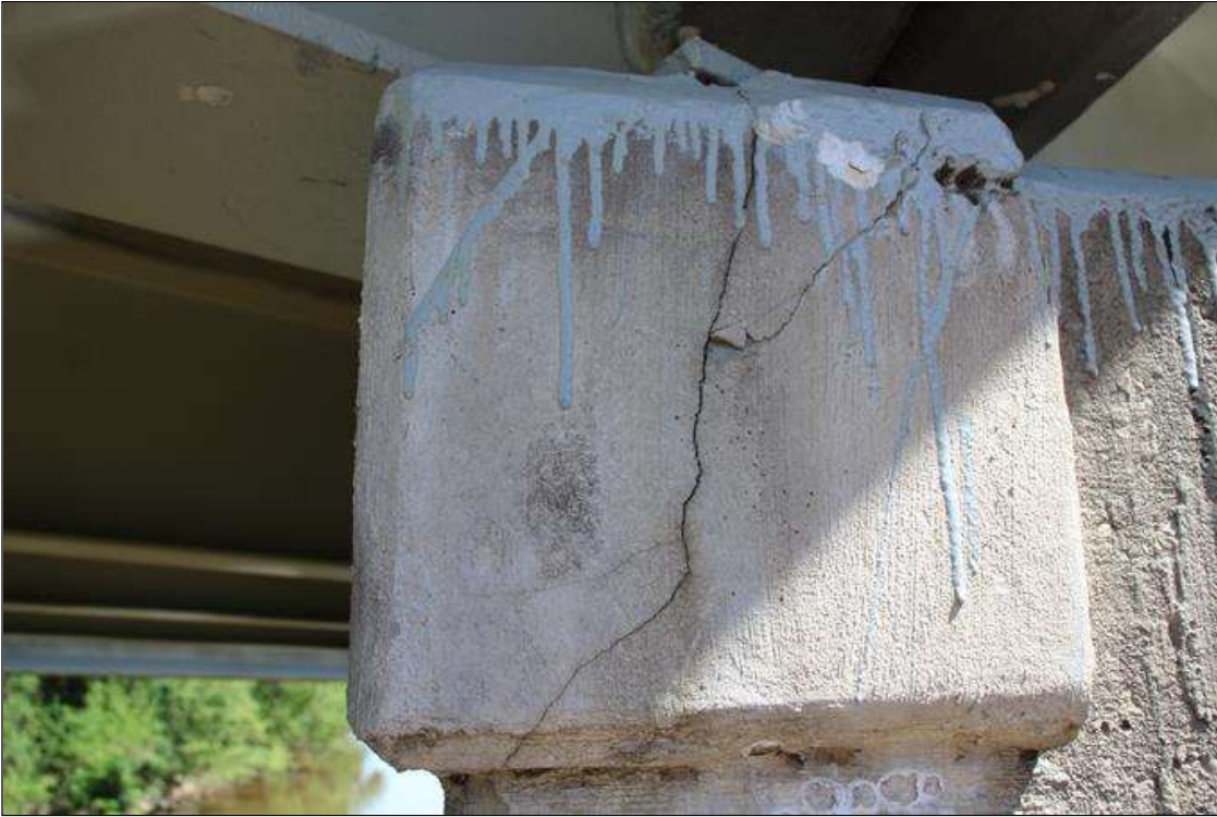
Bent 4 Cap 1: 15 IN HIGH X 21 IN WIDE SOUND CONCRETE PATCH AREA, TOP SOUTHEAST CORNER OF CAP, BELOW NEW BEARING ASSEMBLY OF BEAM 4. PATCH EXHIBITS A 8 IN LONG X 0.02 IN WIDE DIAGONAL CRACK STARTING AT TOP LEFT CORNER IN SOUTH FACE AND A UP TO 0.03 IN WIDE X 15 IN LONG VERTICAL CRACK IN EAST FACE.
