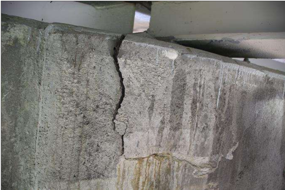
Bent 4 Cap 1: UP TO 2 FT DIAMETER UNSOUND CONCRETE PATCH REPAIR TO PREVIOUSLY SPALLED AREA. PHOTO TAKEN BEFORE AREA WAS SOUNDED WITH HAMMER.
