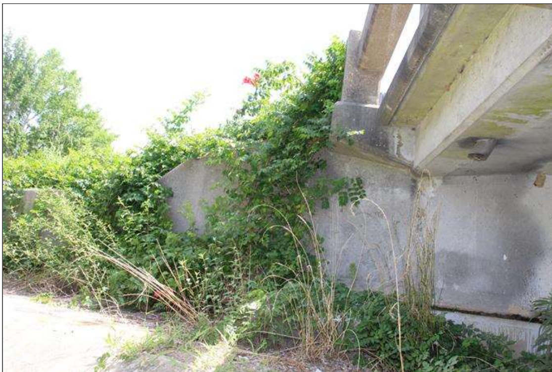
NORTHWEST WINGWALL. NOTE HEAVY VEGETATION.
