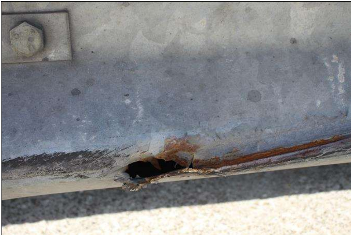
Span 8 Right Bridge Rail: HEAVY IMPACT DAMAGE WITH UP TO 3 IN LONG X 1 IN HIGH HOLES AND DENTS IN THE BOTTOM OF CONCRETE SUPPLMENTAL BRIDGE RAIL FOR FULL SPAN LENGTH. DAMAGE EXTENDS INTO SPANS 7 AND 6.
