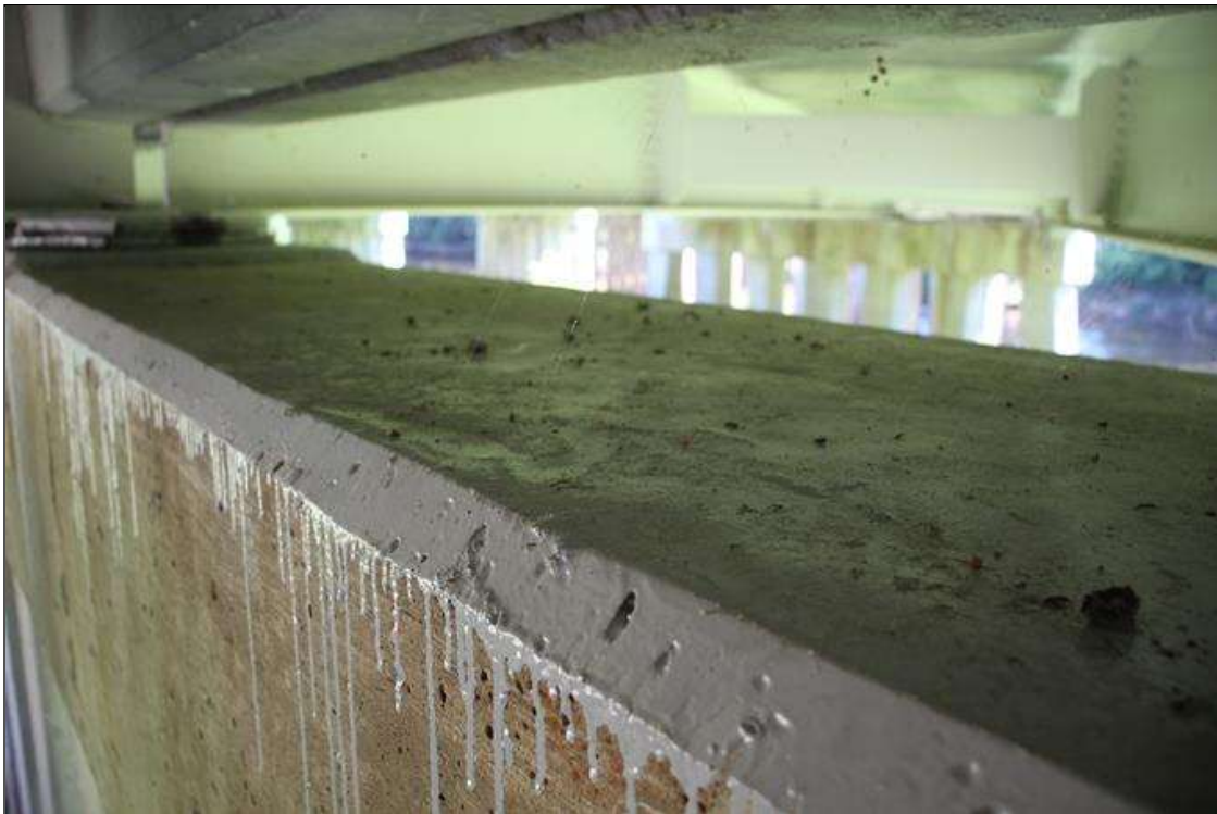
NEW CAP SEAL AT BENT 1 SINCE PREVIOUS INSPECTION. TYPICAL AT ALL BENTS AND END BENTS. BENT 1 BAY 3 SHOWN IN PHOTO.
