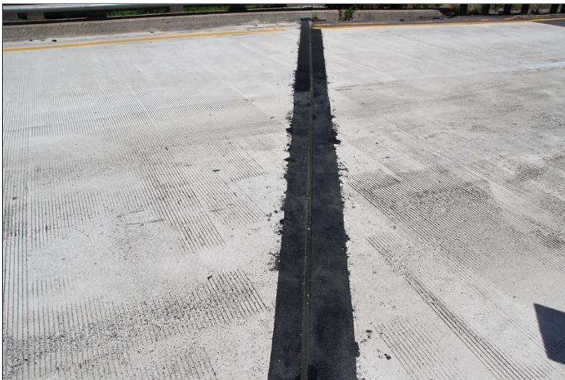
DECK JOINT AT END BENT 2. TYPICAL AT ALL BENTS. NEW SINCE PREVIOUS INSPECTION.
