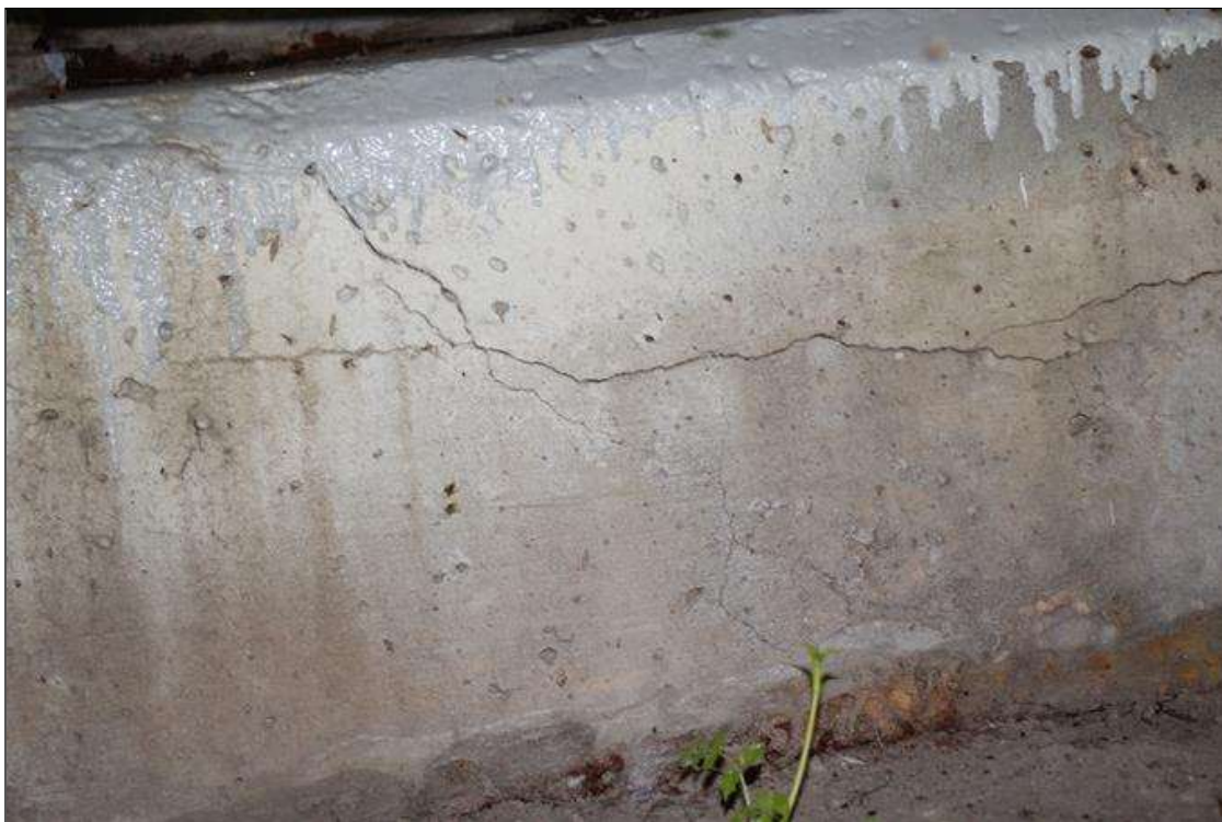
End Bent 2 Abutment/Backwall : UP TO 1/16 IN WIDE X 15 FT LONG HORIZONTAL CRACK IN BAYS 1 AND 2.
