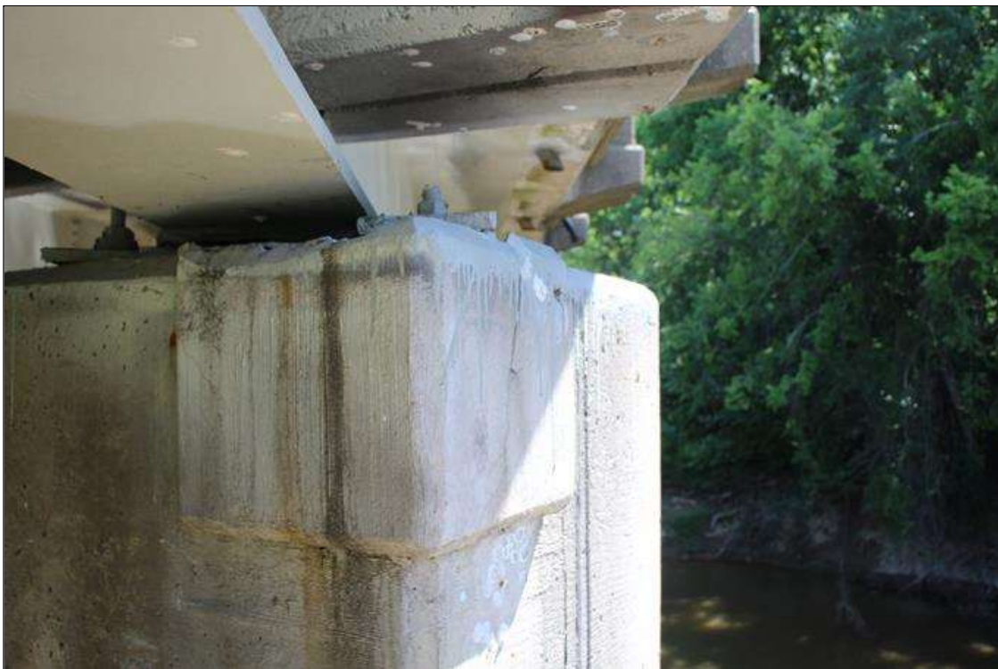
Bent 4 Cap 1: 15 IN HIGH X 21 IN WIDE SOUND CONCRETE PATCH AREA, TOP SOUTHEAST CORNER OF CAP, BELOW NEW BEARING ASSEMBLY OF BEAM 4. PATCH EXHIBITS A 8 IN LONG X 0.02 IN WIDE DIAGONAL CRACK STARTING AT TOP LEFT CORNER IN SOUTH FACE AND A UP TO 0.03 IN WIDE X 15 IN LONG VERTICAL CRACK IN EAST FACE.
