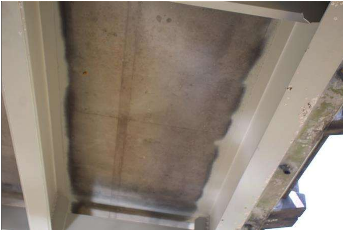
TPYICAL DECK UNDERSIDE SPAN 5 BAY 1. NOTE NEW DECK SINCE PREVIOUS INSPECTION.
