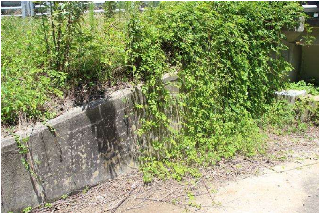
SOUTHEAST WINGWALL. NOTE HEAVY VEGETATION.
