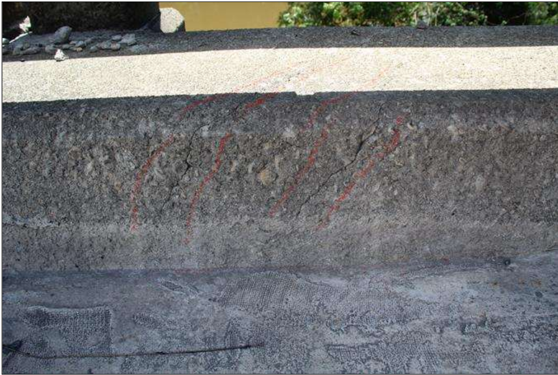
Span 2 Right Bridge Rail: UP TO 0.03 IN WIDE X 2 FT LONG DIAGONAL CRACKS IN BOTTOM OF CURB AT 1 FT FROM BENT 2.
