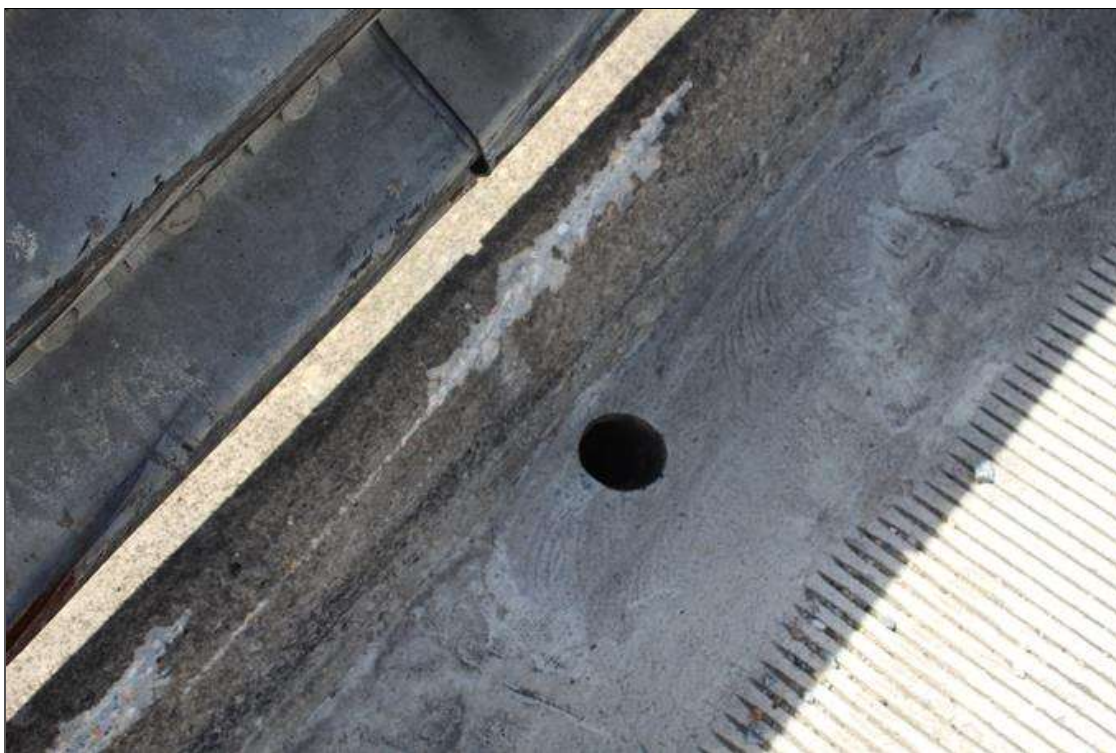
DECK DRAIN ALONG LEFT BRIDGE RAIL IN SPAN 8. TYPICAL ALONG BOTH BRIDGE RAILS IN ALL SPANS.
