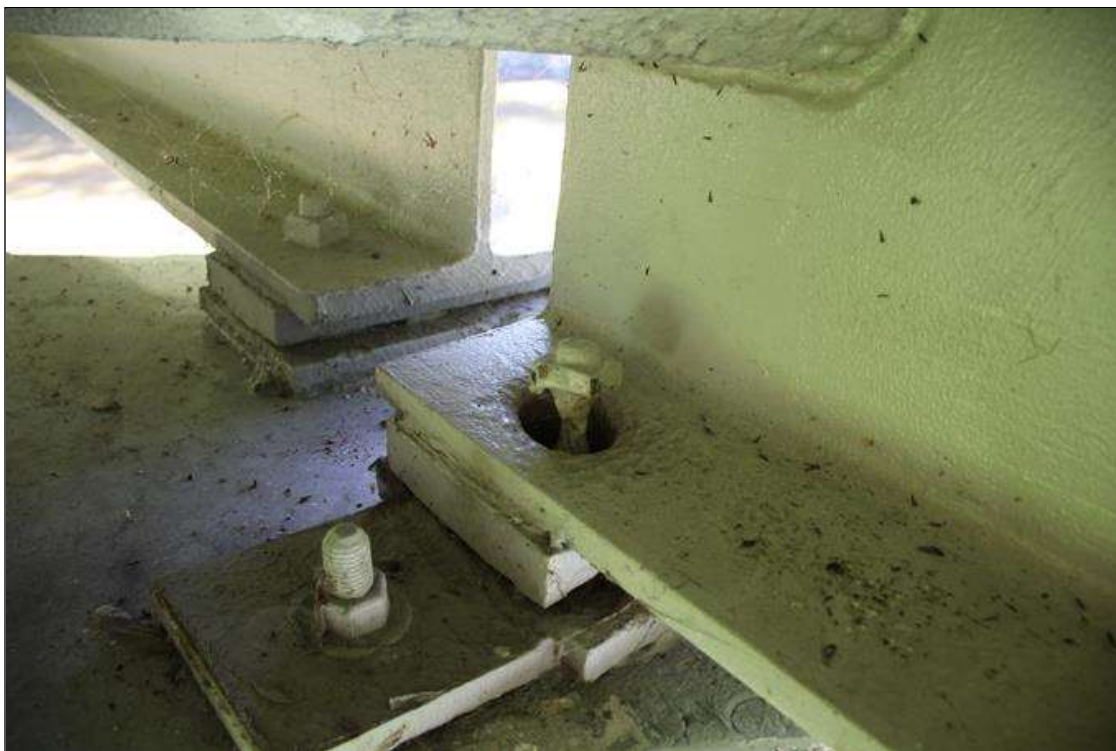
Span 2 Beam 4 Far Bearing: WELDED REPAIR WITH NEW ANCHOR BOLT. UP TO 50% SECTION LOSS IN OLD ANCHOR BOLT. PAR NOT ISSUED DUE TO NEW ANCHOR BOLT REPAIR.
