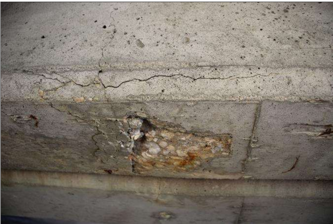
Span 5 Deck: 6 IN DIAMETER X 3/4 IN DEEP SPALL IN INTERMEDIATE DIAPHRAGM IN BAY 2 ABOVE BENT 6.
