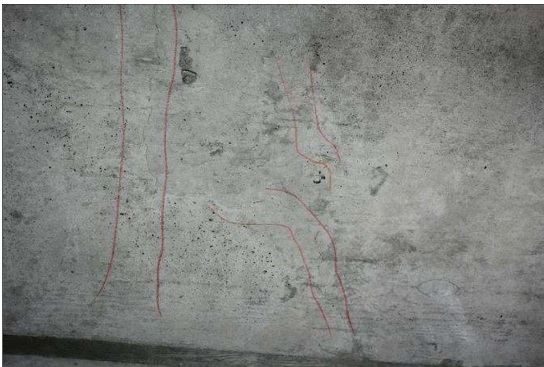
Span 1 Deck: UP TO 0.02 IN WIDE TRANSVERSE CRACKS IN DECK UNDERSIDE IN BAY 1 BETWEEN INTERMEDIATE DIAPHRAGMS TYPICAL IN BAYS 2 AND 3.
