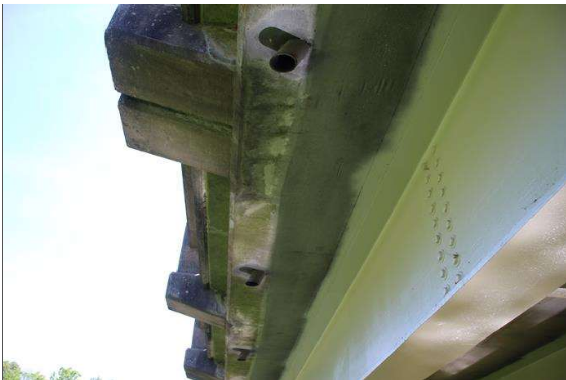
DECK DRAINS UNDER LEFT OVERHANG IN SPAN 3. TYPICAL ALONG BOTH BRIDGE RAILS IN ALL SPANS.
