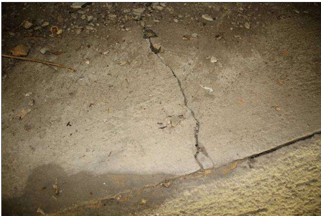
End Bent 2 Cap 1: 3 FT LONG X UP TO 1/16 IN WIDE HORIZONTAL CRACK, BELOW BAY 1.
