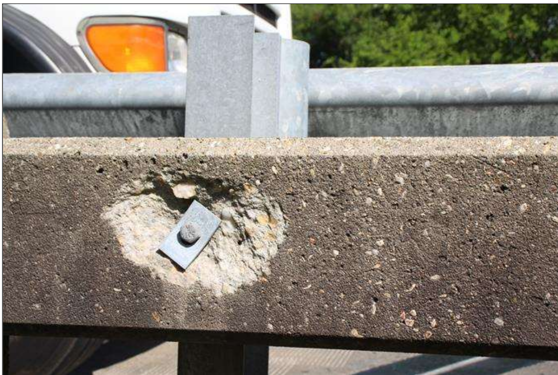
Span 2 Right Bridge Rail: UP TO 6 IN DIAMETER X 1.5 IN DEEP SPALL IN EXTERIOR FACE AT ANCHOR BOLT CONNECTION. TYPICAL AT SEVERAL CONNECTIONS.
