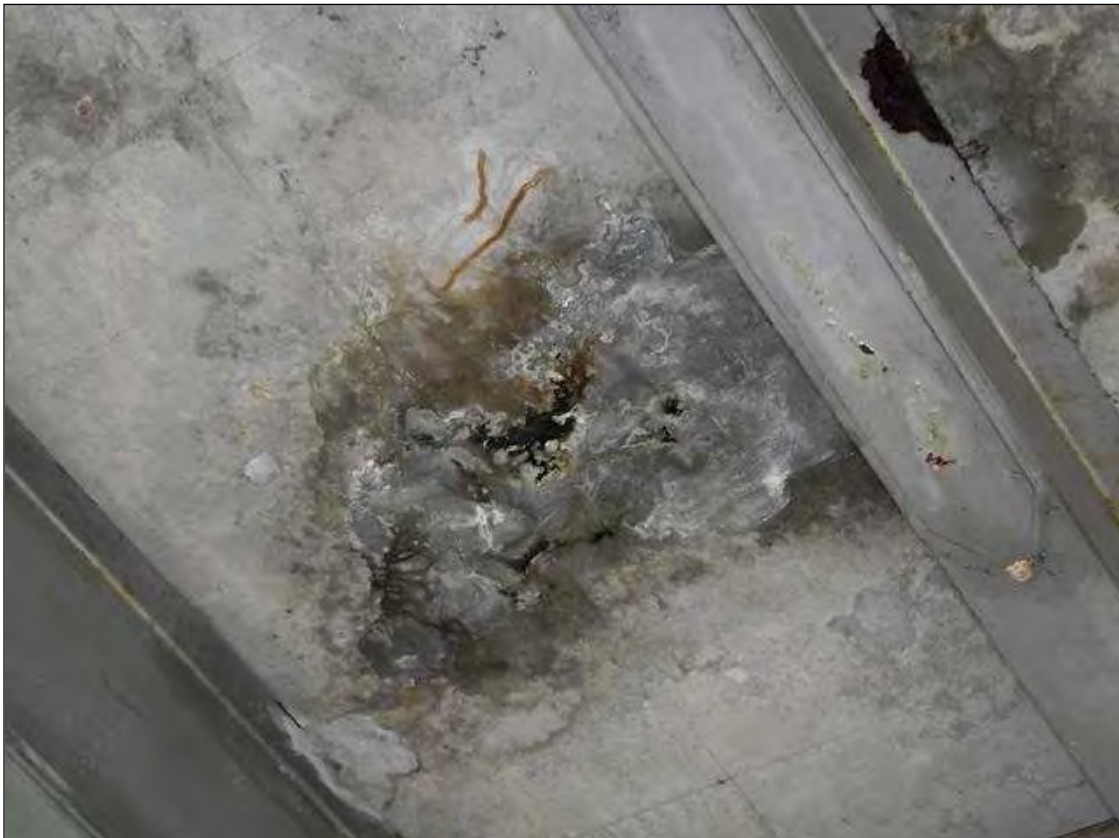
AREA OF MAP CRACKING WITH EFFLORESCENCE IN BOTTOM OF DECK OF SPAN 7 BAY 2 BETWEEN INTERIOR DIAPHRAGMS
