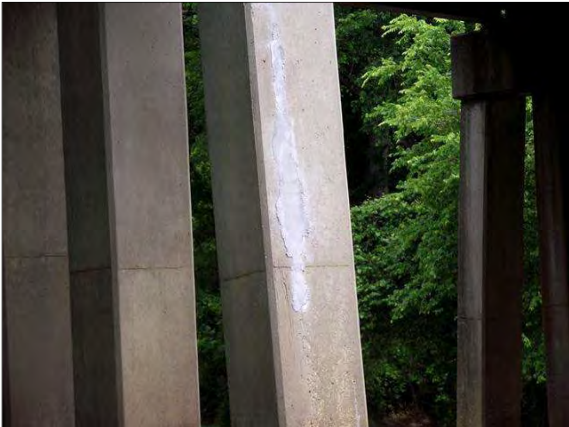
REPAIR PATCH IN THE RIGHT SIDE FACE OF PILE 7 AT BENT 3
