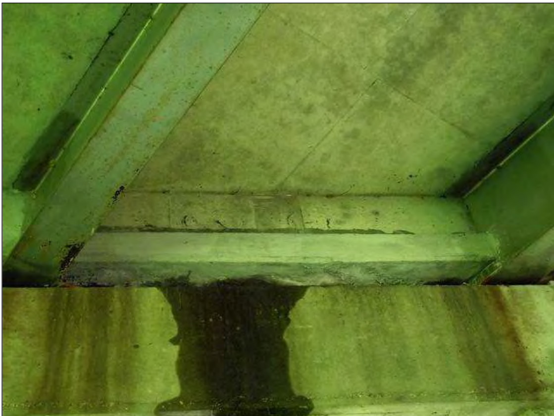
SPALL REPAIR IN SPAN 2 END DIAPHRAGM AT BENT 2 BAY 2 - BAY 3 SIMILAR
