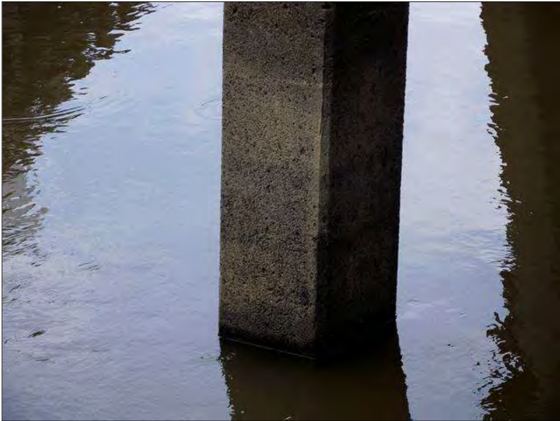
ABRASION WITH EXPOSED COARSE AGGREGATE IN FACES OF PILES IN WATERWAY
