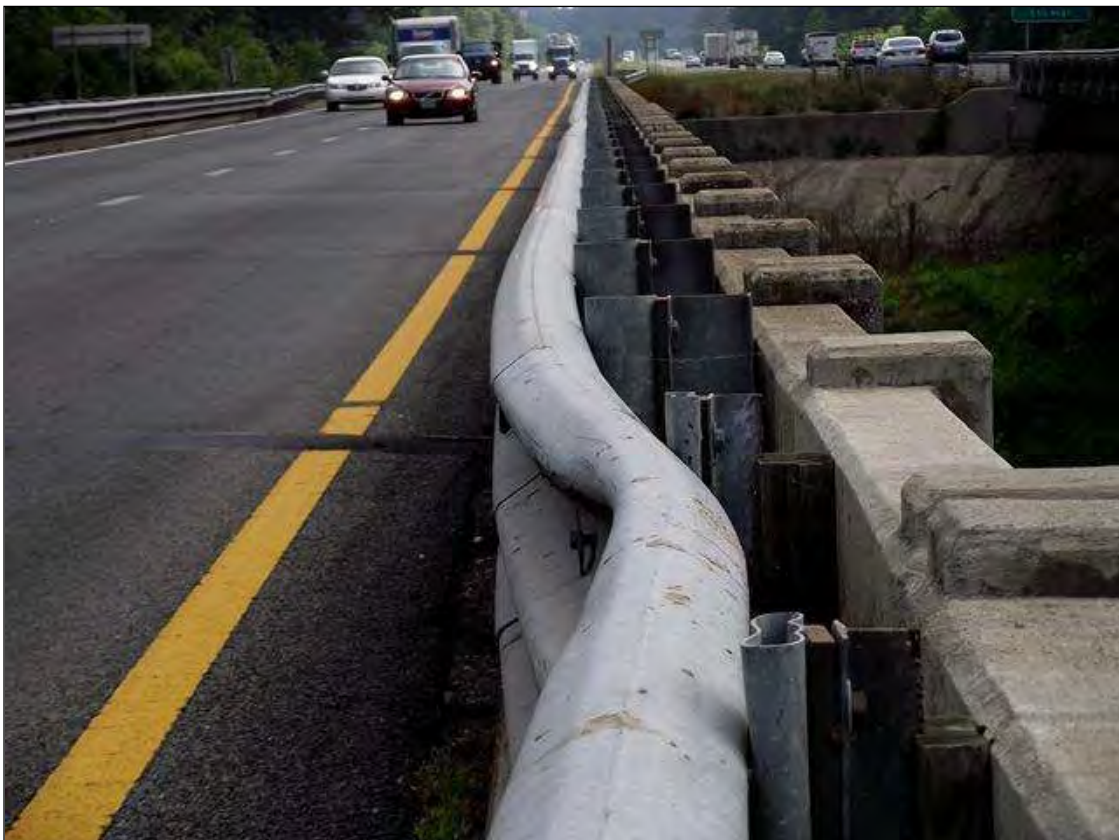
IMPACT DAMAGE TO THE RIGHT SIDE GUARDRAIL IN SPAN 1
