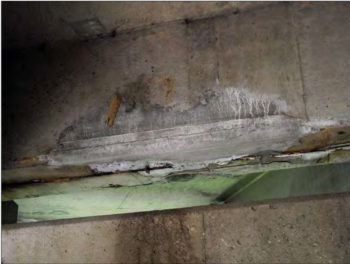
SPALL REPAIR IN SPAN 8 END DIAPHRAGM AT BENT 7 BAY 2
