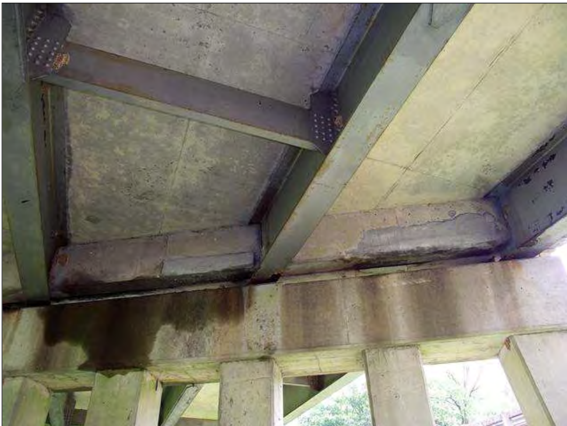
SPAN 1 END DIAPHRAGMS PATCHED AT BENT 1 BAYS 2 & 3
