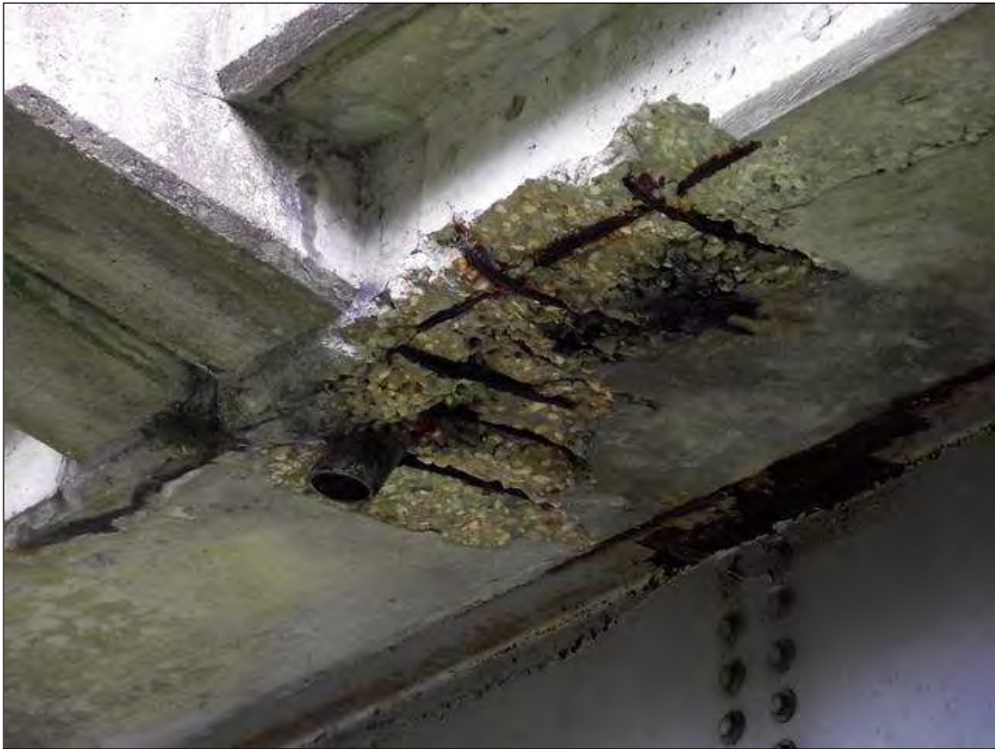
SPALLED AREA WITH SECTION LOSS TO EXPOSED REBAR IN THE RIGHT SIDE OVERHANG OF SPAN 7 AT 1/3 POINT FROM BENT 6
