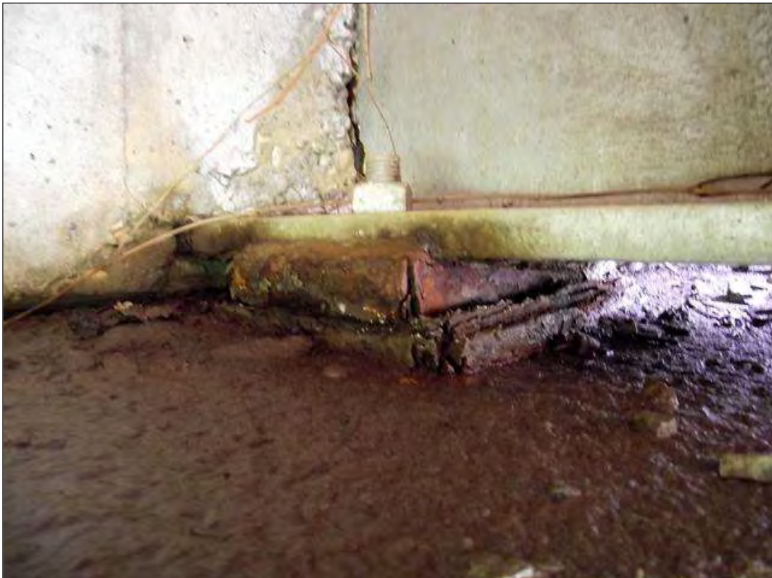
EXTERIOR BEARING ASSEMBLIES AT END BENT 2 ARE RUSTY AND FLAKING
