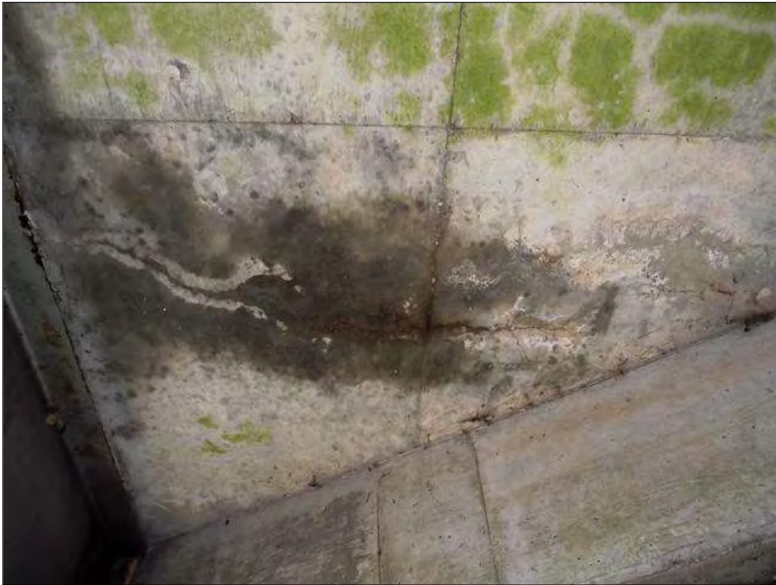
HAIRLINE DIAGONAL CRACK WITH EFFLORESCENCE IN BOTTOM OF DECK OF SPAN 8 BAY 3 NEAR BENT 7
