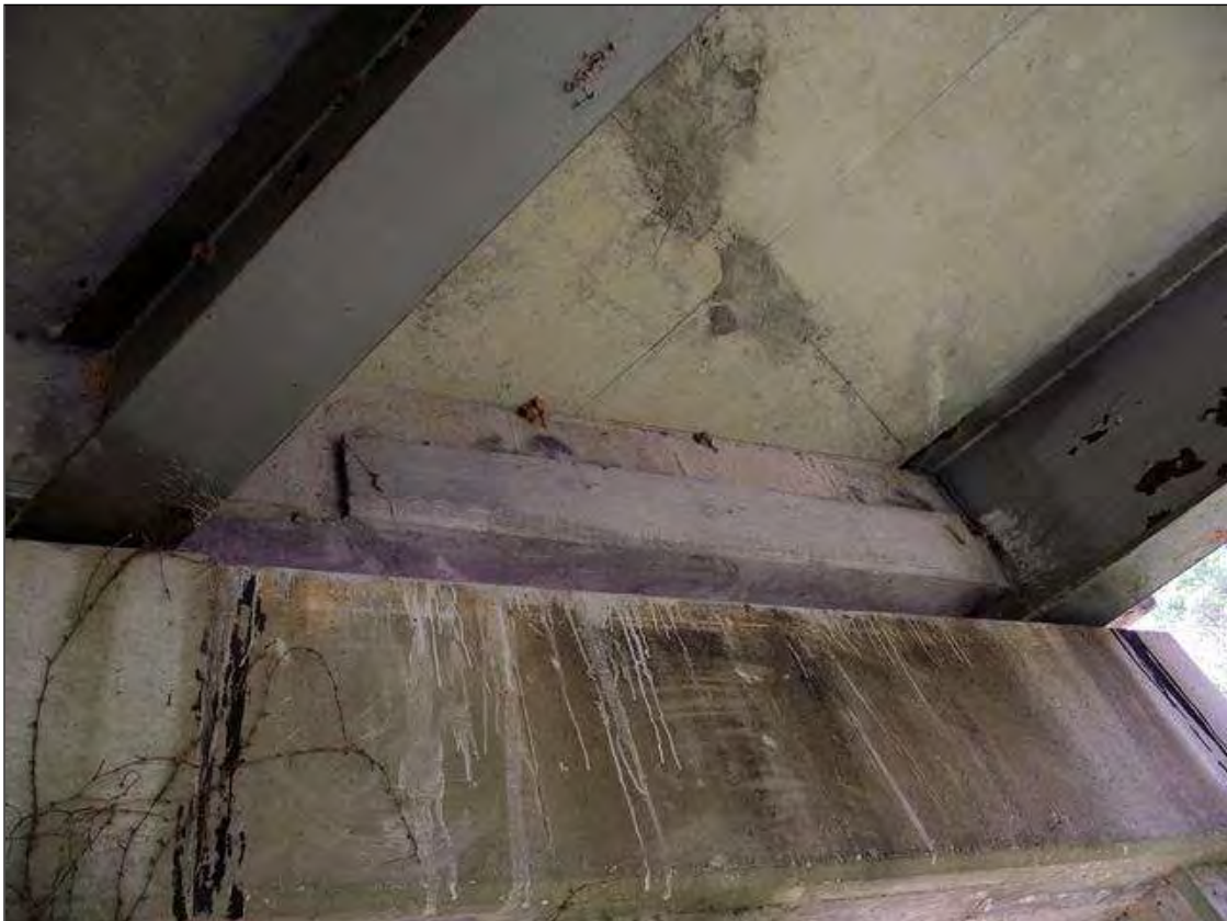
SPALL REPAIR IN SPAN 7 END DIAPHRAGM AT BENT 7 BAY 3
