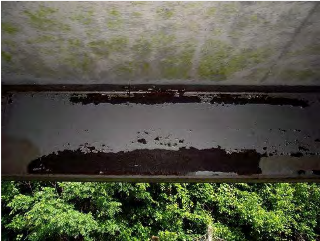
RANDOM AREAS OF PEELING PAINT & SURFACE RUST IN BEAM WEBS THROUGHOUT STRUCTURE
