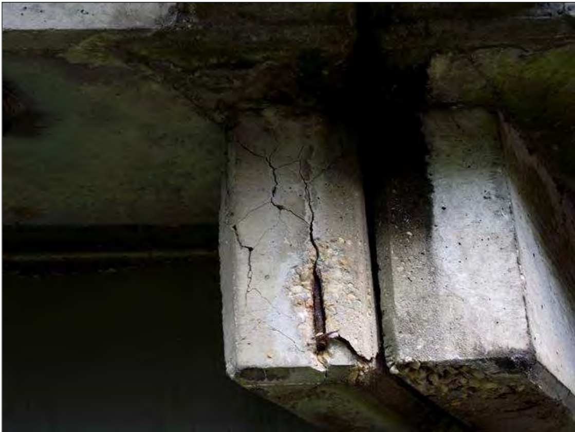
CRACKED AND SPALLED AREA WITH EXPOSED REBAR THE RIGHT EXTERIOR DIAPHRAGM OF SPAN 7 AT BENT 7
