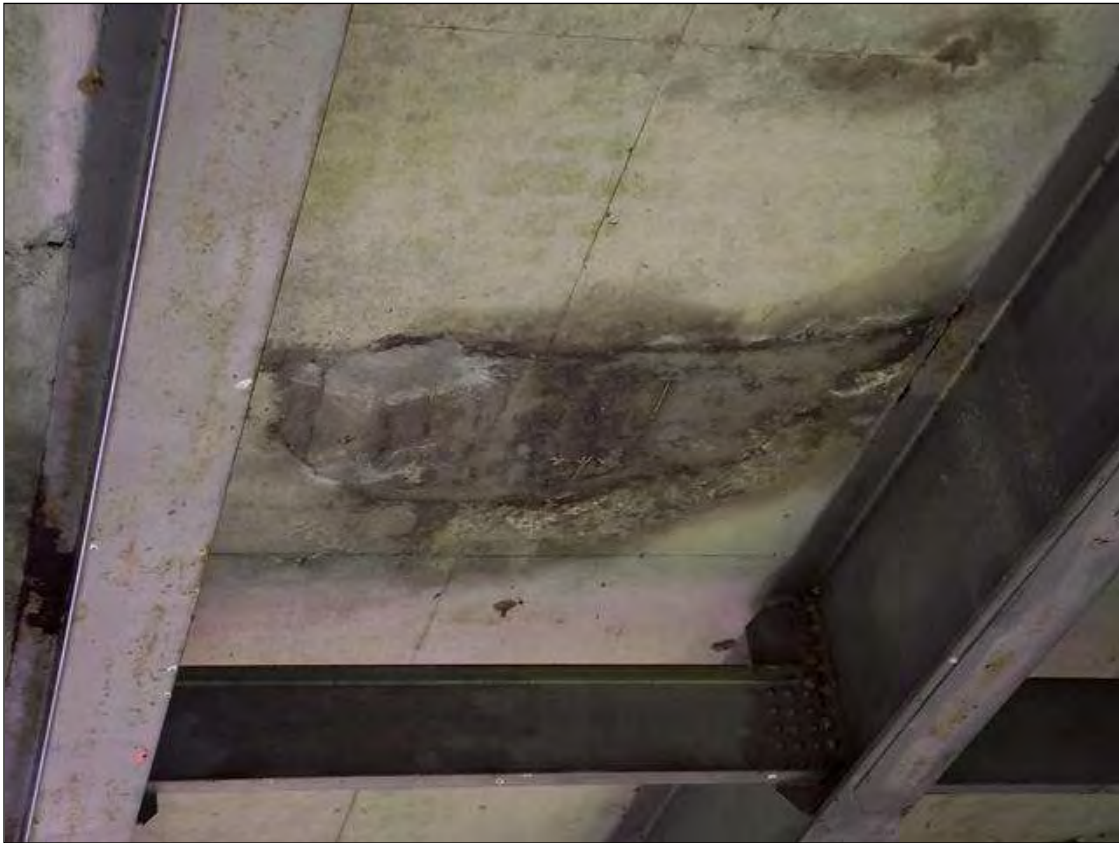
REPAIR PATCHES IN BOTTOM OF DECK OF SPAN 7 BAY 3 AT 1/3 POINT - SIMILAR PATCHES THROUGHOUT SPAN
