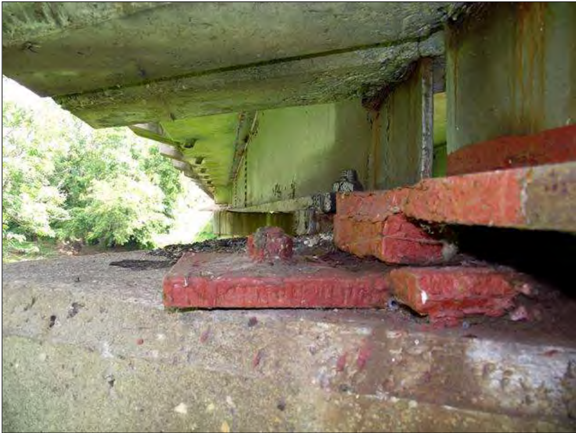
ANCHOR BOLT REPAIR FOR BEAM 1 AT BENT 1 (PLATES ADDED ADJACENT TO BEARING ASSEMBLIES) - OTHER REPAIRS SIMILAR THROUGHOUT STRUCTURE
