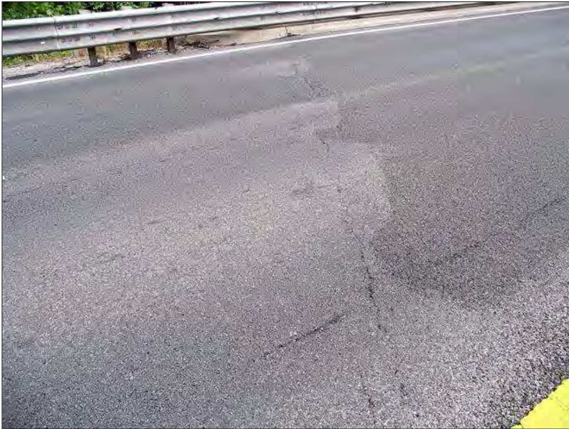
TRANSVERSE CRACK IN WEARING SURFACE OVER END BENT 1
