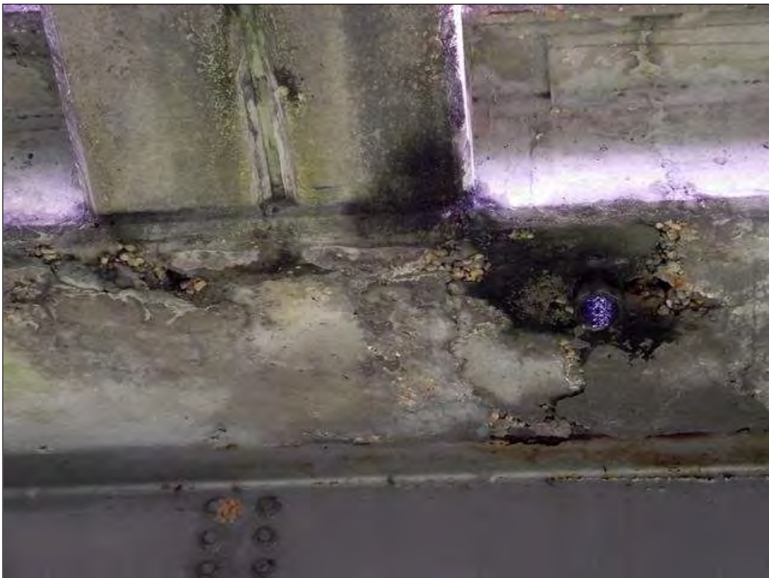
CRACKED AND DELAMINATED AREA IN THE RIGHT SIDE OVERHANG OF SPAN 7 AT MID-SPAN
