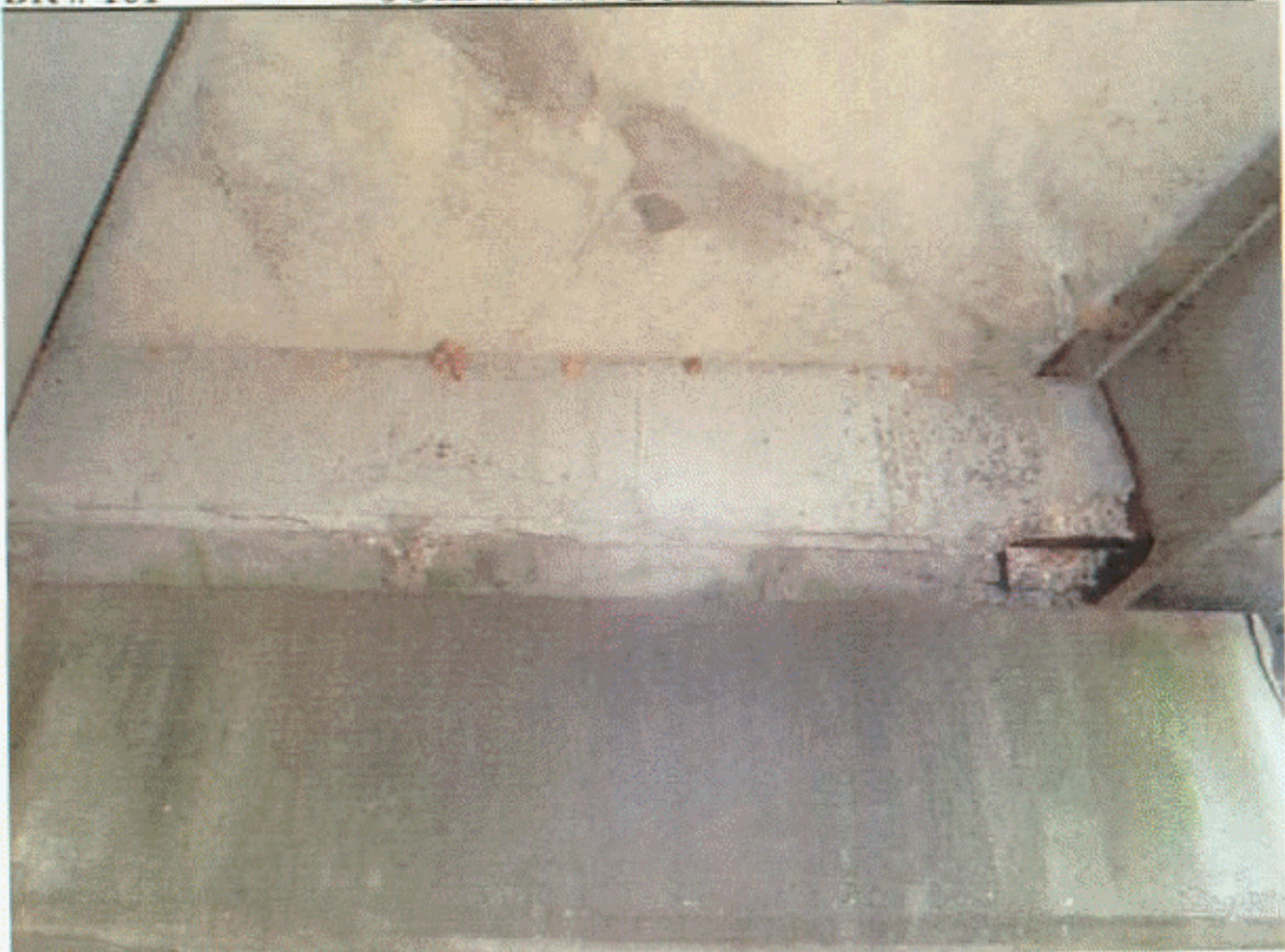
BT-7, SP-7; DIAPH SPALLED LT OF BM-4, ALSO CRKD AND DELAM
