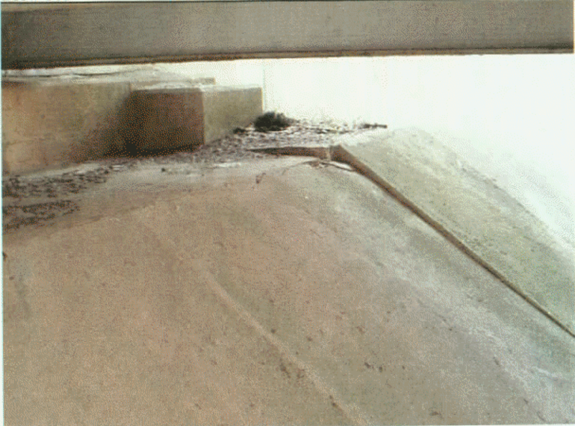
SLOPE PROTECTION CRKD AND SETTLED IN SP-1
