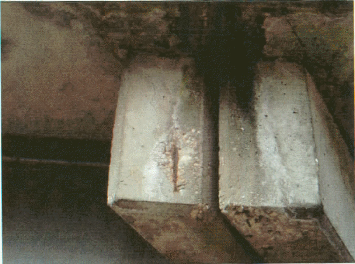
BT-7, SP-7; RT EXTERIOR DIAPH CRKD AND SPALLED
