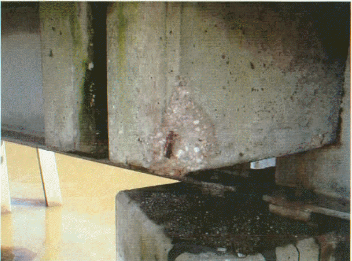
BT-3, SP-3; LT EXTERIOR DIAPH SPALLED
