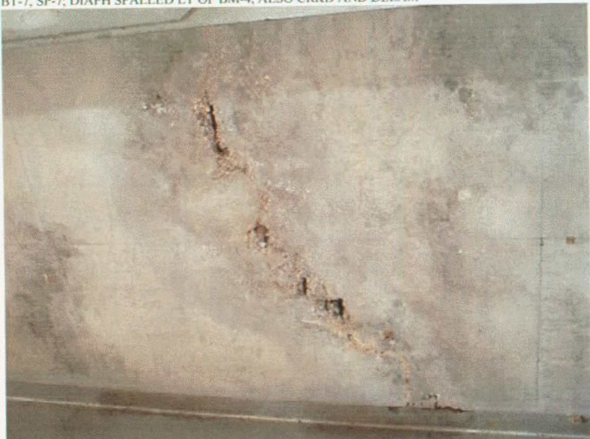
SP-7 @ .6 PT, HONEYCOMB OVER EXPOSED REBARS W/ TRANSV CRKNG
