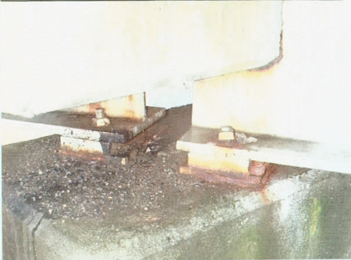
BT-5, SP-5, BM-1 BRNG IS HEAVILY RUSTED (MOST OTHERS SIMILAR)
