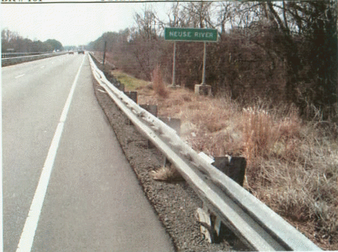
NW APPROACH RAIL DAMAGED
