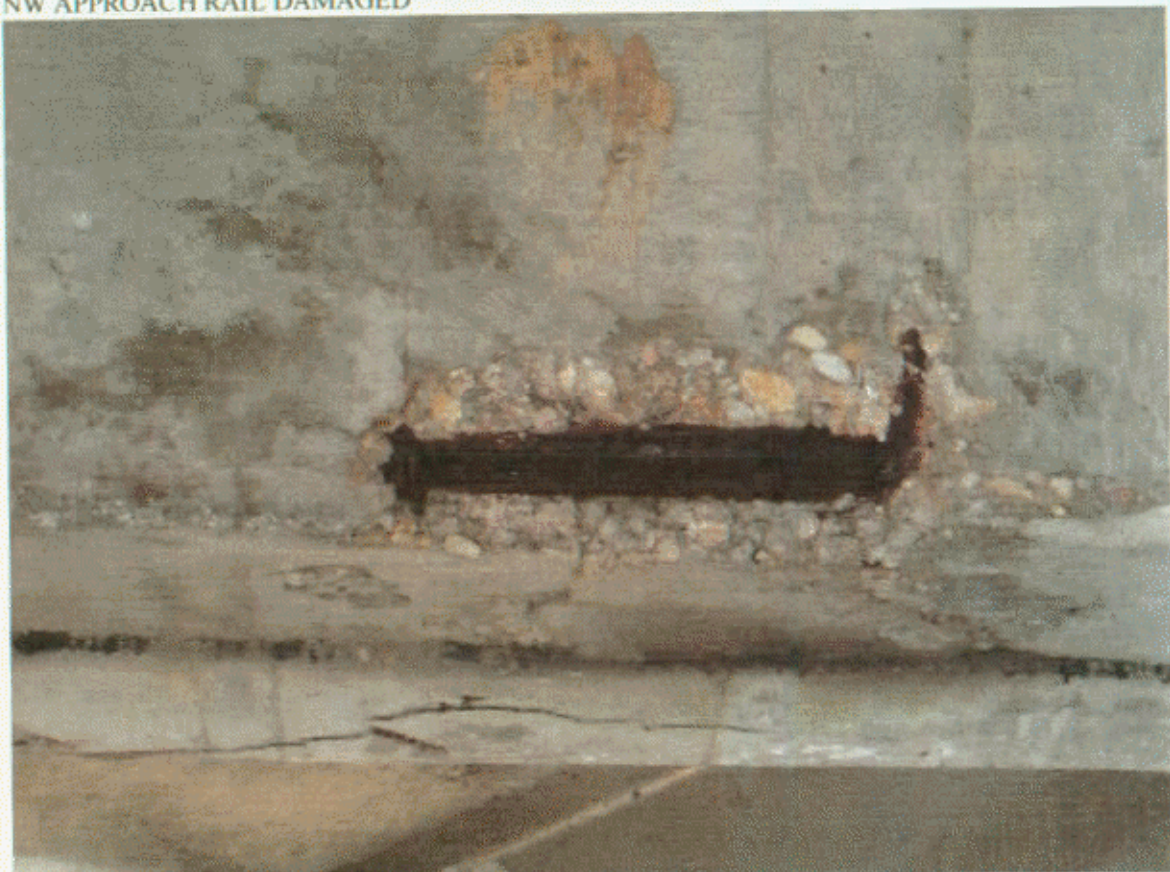
BT-7, SP-8; BAY-2 DIAPH SPALLED W/ REBAR EXPOSED (ALSO CRKD ON SP-7 SIDE)
