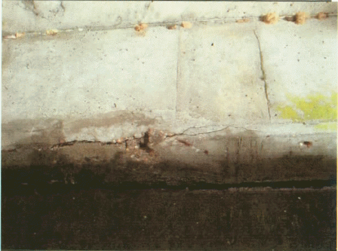
BT-4, SP-4, BAY-1 DIAPH CRKD AND SPALLED
