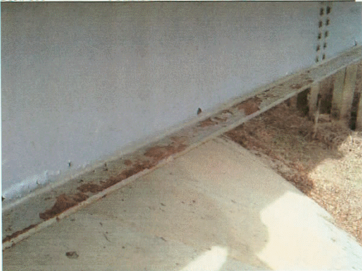
BM-4, SP-1, TOP FLANGE RUSTING (ALL EXTERIOR BMS SIMILAR)
