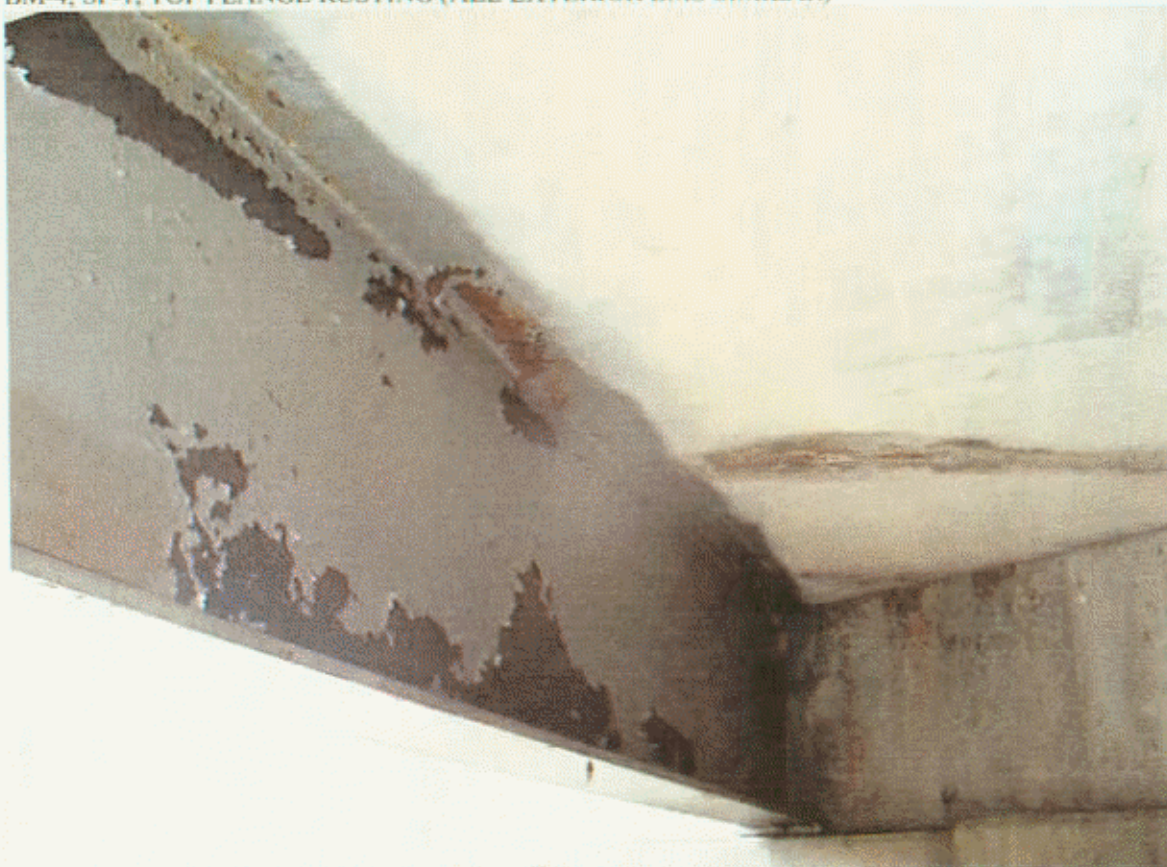
BM-4, SP-1; PAINT PEELING & DIAG CRK IN BOD W/ RUST AND EFFLO IN BAY-3
