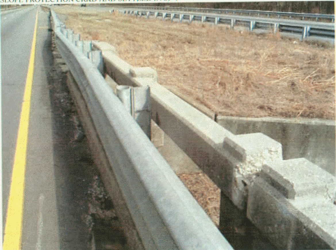
RT RAIL CONC. SPALLED W/ METAL RAIL DAMAGED
