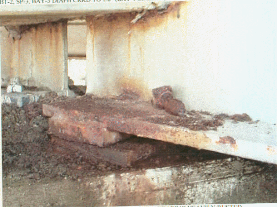
BT-2, SP-2, BM-1 LT ANCHOR BOLT RUSTED INTO & BEARING HEAVILY RUSTED
