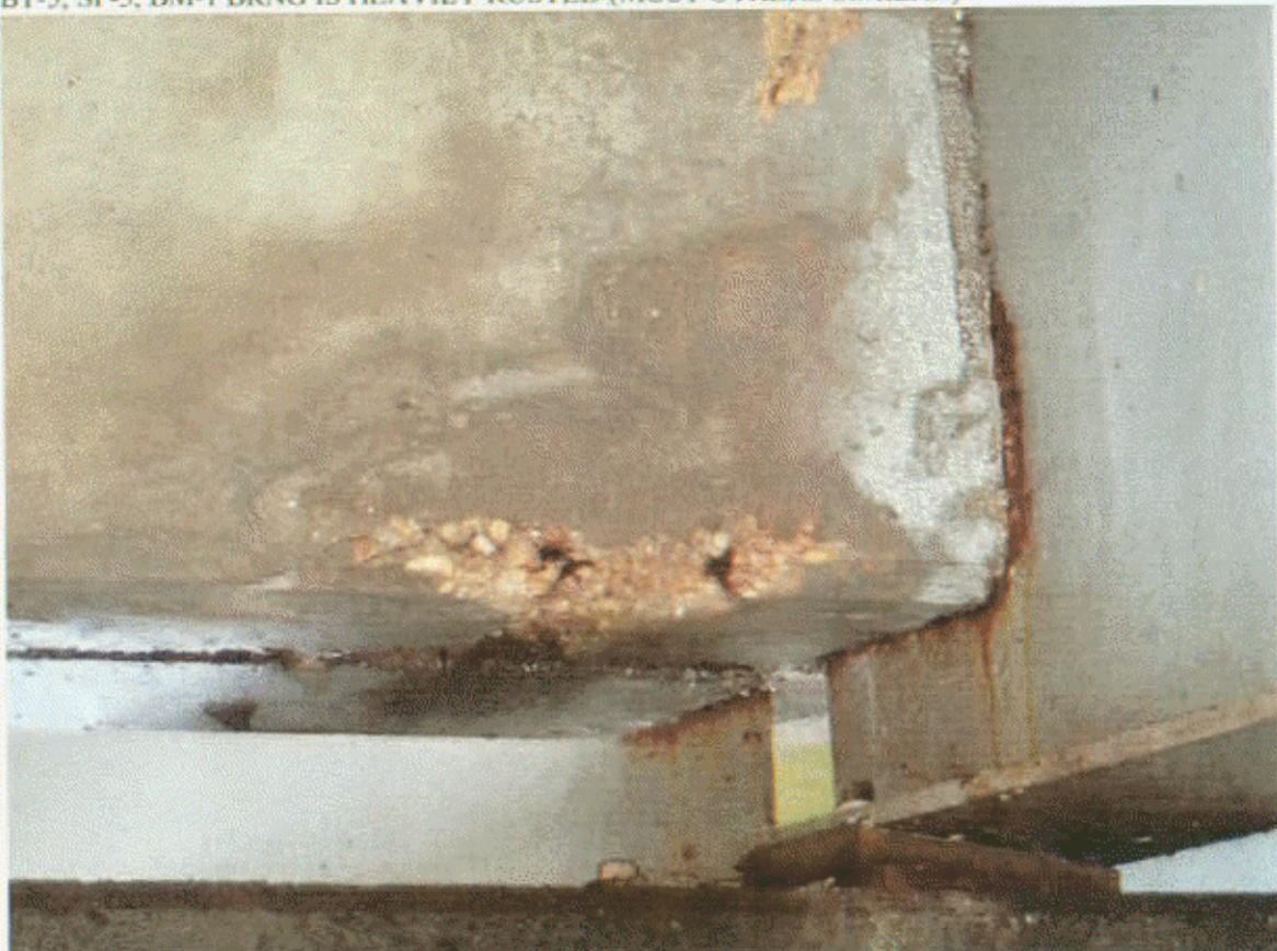
BT-4, SP-5, BAY-2 DIAPH SPALLED RT OF BM-2
