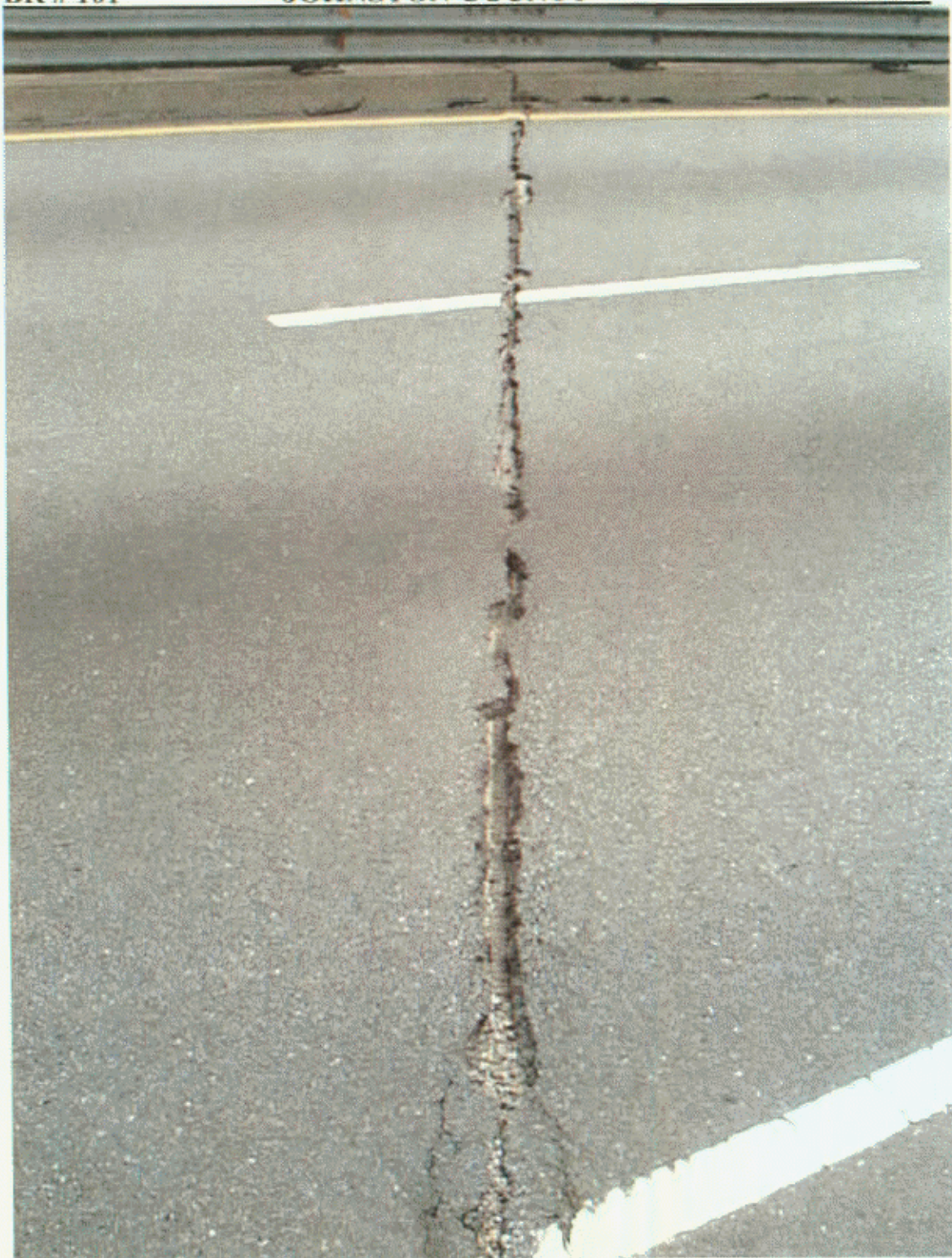
AWS CRKD OR MISSING ALONG JOINT AT BT-1
