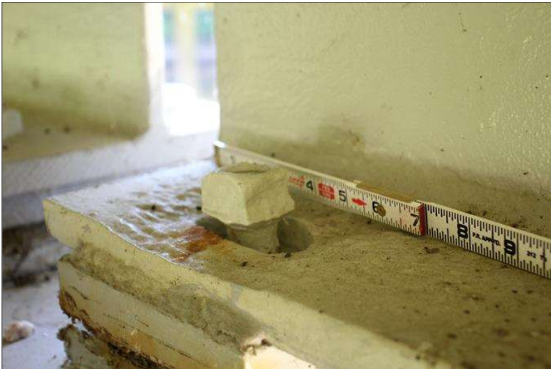
Span 1 Beam 4: 5 IN LONG X 5 IN WIDE AREA OF HEAVY SURFACE CORROSION BENEATH THE PAINTED SURFACES IN BOTTOM FLANGE OF LEFT FLANGE ABOVE BEARING AT BENT 1. UP TO 0.8 IN SECTION REMAINING.
