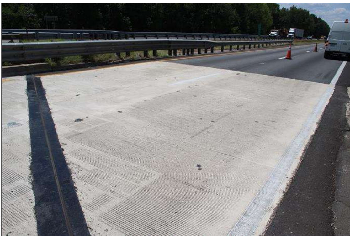
SOUTH APPROACH SLAB. NEW SINCE PREVIOUS INSPECTION. NOTE NEW ASPHALT PAVEMENT IN SOUTH APPROACH.
