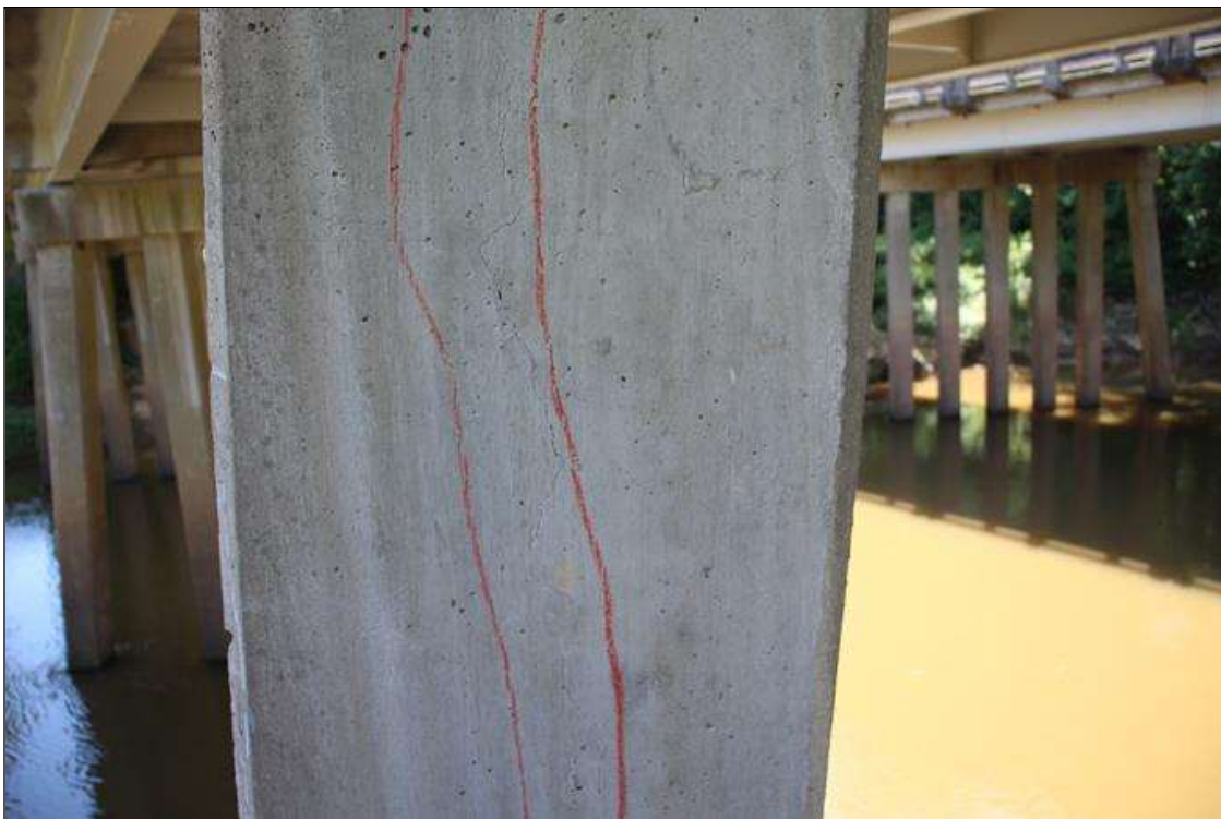
Bent 4 Pile 1: 5 FT LONG X 0.02 IN WIDE VERTICAL CRACK, SOUTH FACE BEGINNING AT CAP.
