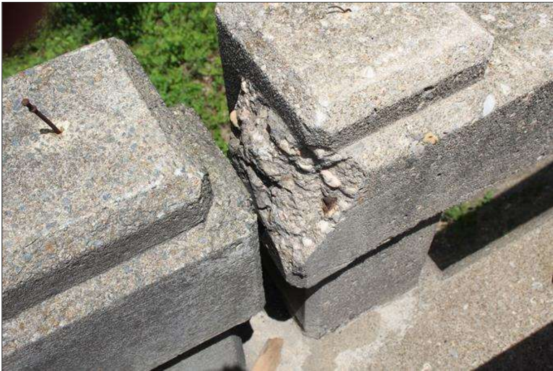
Span 8 Left Bridge Rail: 8 IN WIDE X 8 IN HIGH X UP TO 3 IN DEEP SPALL WITH EXPOSED REINFORCEMENT IN TOP OF RAIL AT FIRST RAIL JOINT FROM END BENT 2. 90% SECTION REMAINING IN EXPOSED REINFORCEMENT.
