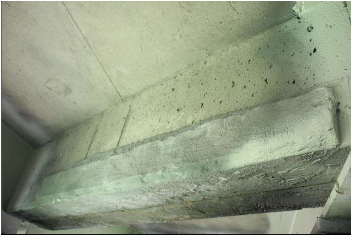
Span 2 Deck: 82 IN WIDE X 1 FT HIGH SOUND CONCRETE PATCH AREA, BAY 2 END DIAPHRAGM, AT BENT 1.
