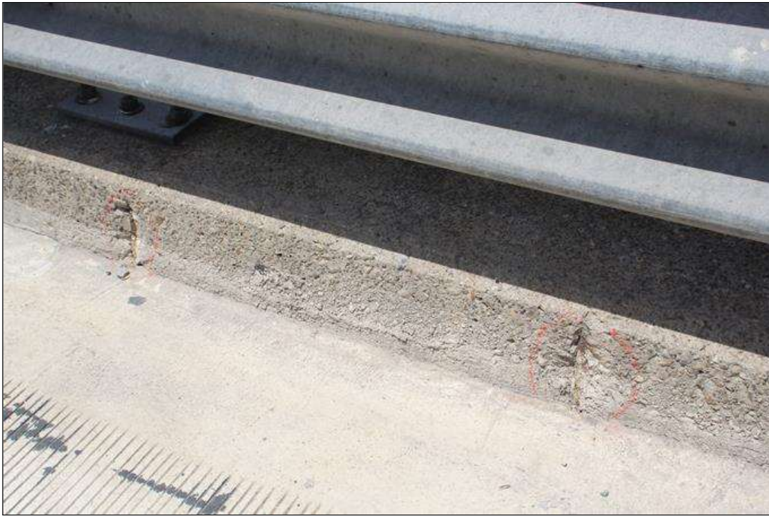
Span 3 Left Bridge Rail: TWO (2) SPALLS UP TO 8 IN IN DIAMETER X 1 IN DEEP WITH EXPOSED REINFORCEMENT IN BOTTOM OF CURB AT 6 FT AND 10 FT FROM BENT 3 JOINT. NO MEASURABLE SECTION LOSS IN EXPOSED REINFORCEMENT.
