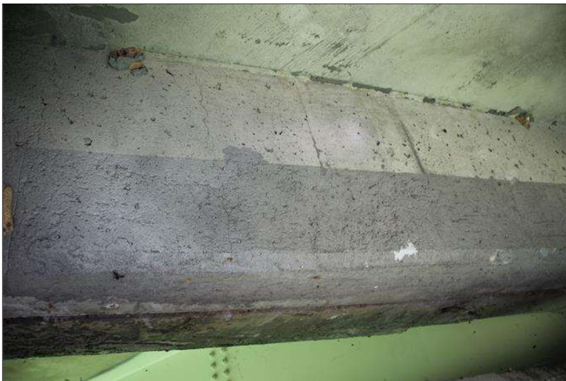
Span 3 Deck: NEW REPAIR: 9 FT LONG X 1 FT HIGH SOUND CONCRETE PATCH IN BAY 3 AT BENT 2.
