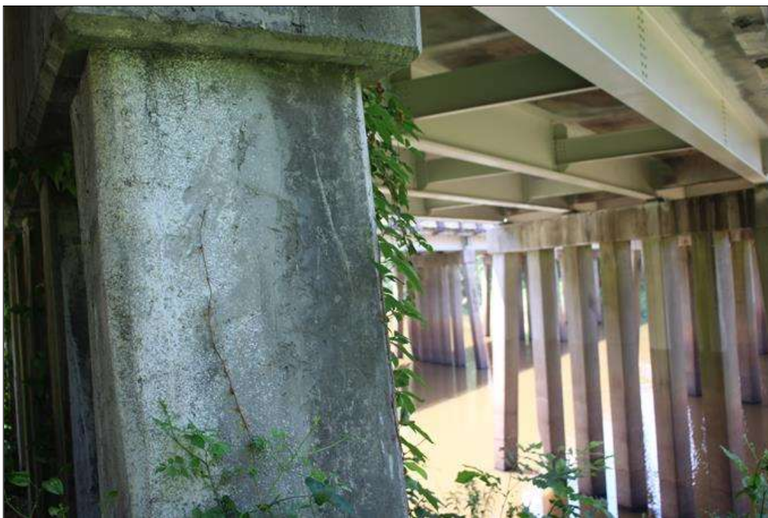
Bent 7 Pile 1: NEW REPAIR 8 FT HIGH X 1 FT WIDE SOUND CONCRETE PATCH IN WEST FACE.
