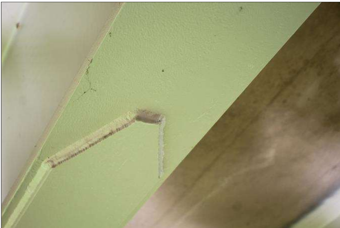
BOTTOM FLANGE COVERPLATE CONNECTION AT BEAM 3 SPAN 3. TYPICAL IN BEAMS 2 AND 3 IN ALL SPANS.
