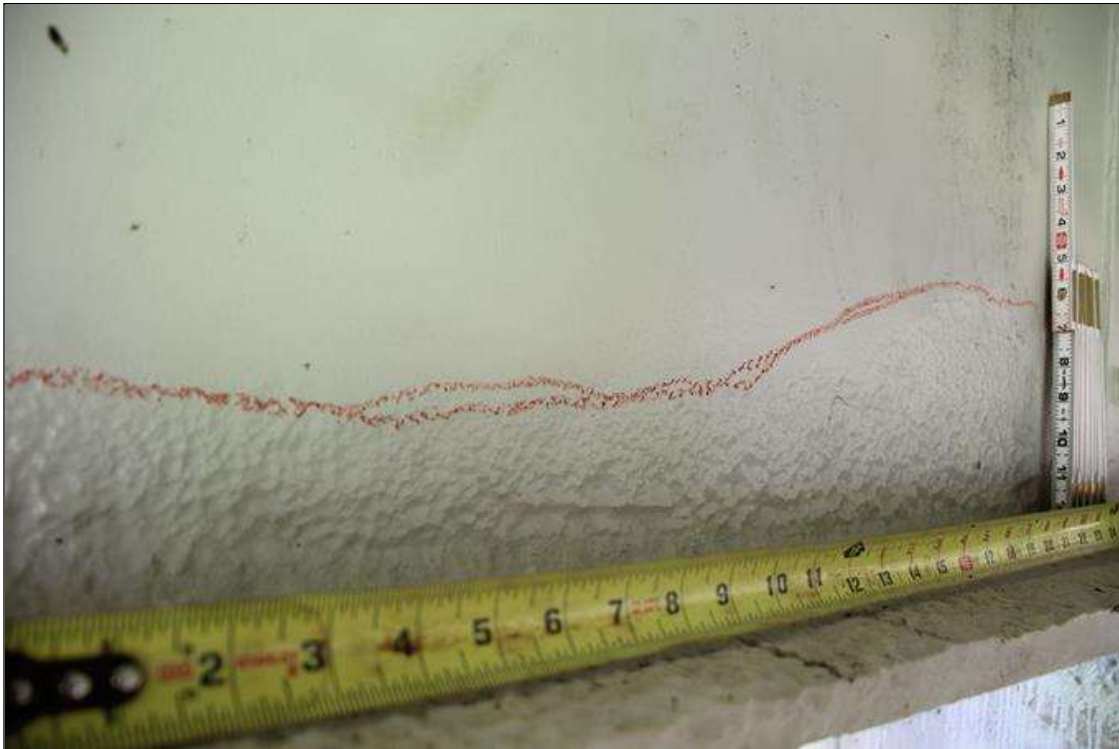
Span 3 Beam 1: 3.3 FT LONG X UP TO 5 IN HIGH AREA OF RIGHT FACE OF THE WEB AT 1.25 FT FROM BEAM END AT BENT 3 EXHIBITS SECTION LOSS BENEATH THE PAINTED SURFACE. UP TO 0.575 IN SECTION REMAINING.
