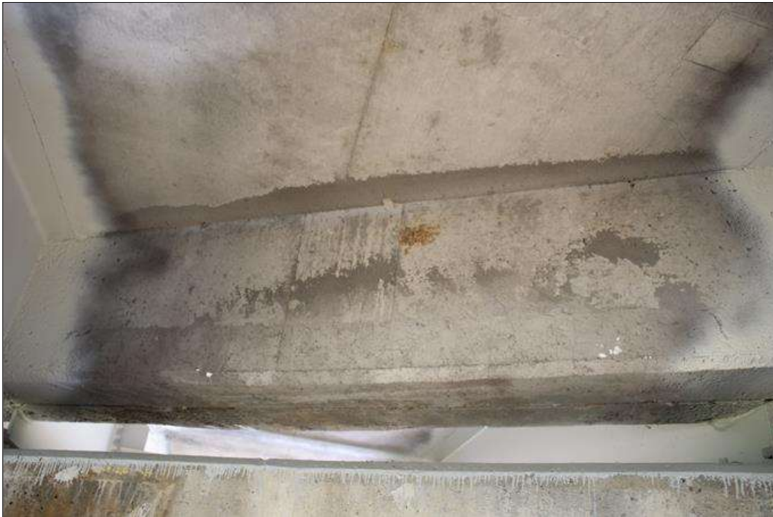
Span 5 Deck: NEW REPAIR: 8 FT LONG X 6 IN HIGH SOUND CONCRETE PATCH IN BAY 2 END DIAPHRAGM, AT BENT 5.
