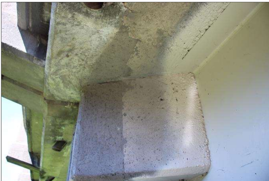
Span 2 Deck: NEW REPAIR: 3 FT WIDE X 1 FT HIGH SOUND CONCRETE PATCH IN OVERHANG IN EAST FACE AT BENT 2 AND A 1 FT WIDE X 2 FT HIGH SOUND CONCRETE PATCH IN DIAPHRAGM OUTSIDE OF BEAM 4 AT BENT 2.
