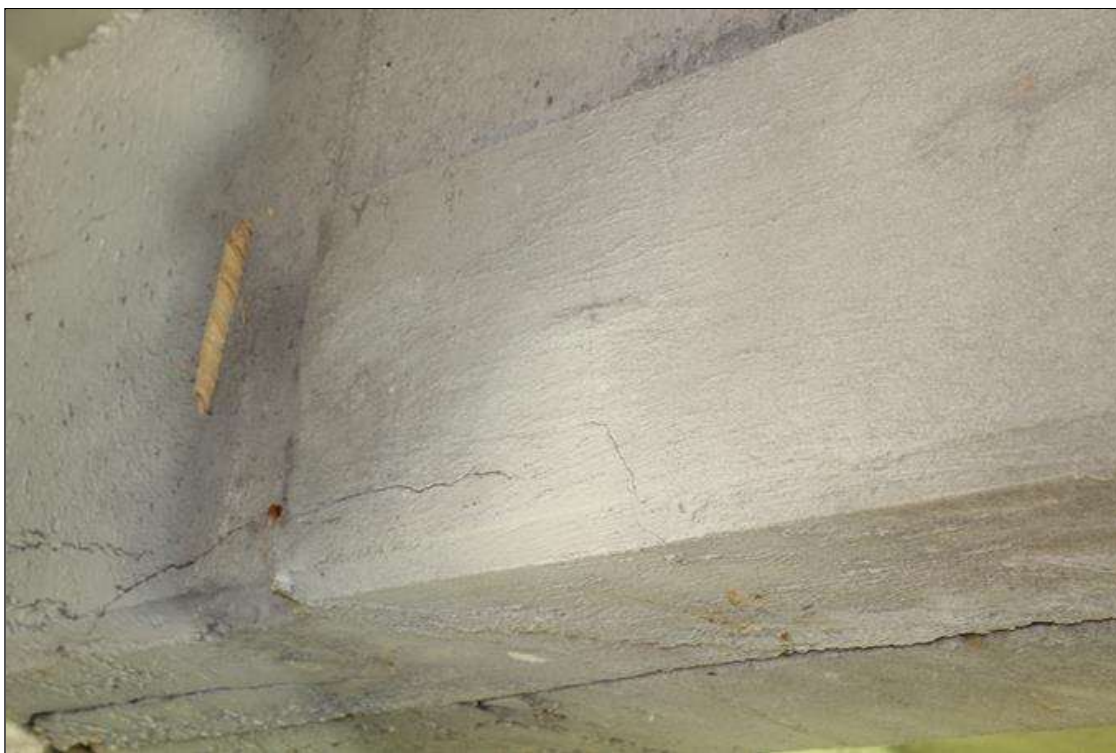
Span 7 Deck: 7 FT LONG X 1 FT HIGH SOUND CONCRETE PATCH IN INTERMEDIATE DIAPHRAGM IN BAY 3 AT BENT 7.
