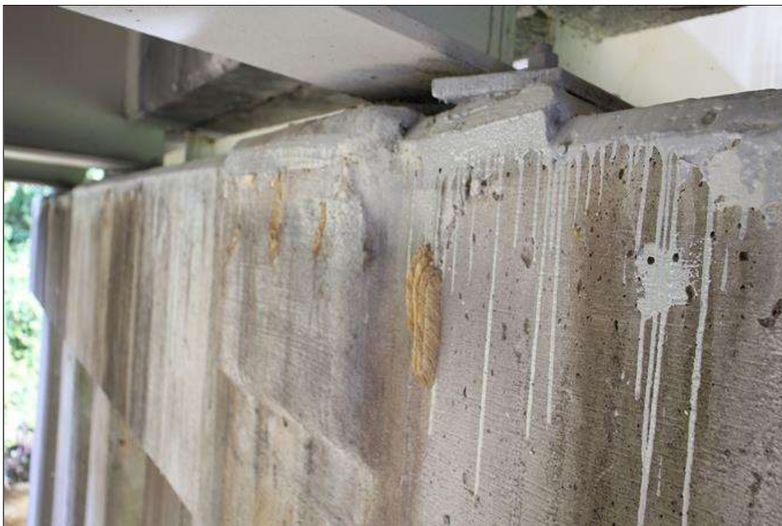
Bent 6 Cap 1: 2 FT LONG X 17 IN HIGH PATCHED AREA, TOP OF SOUTH FACE, BELOW BEAM 3.
