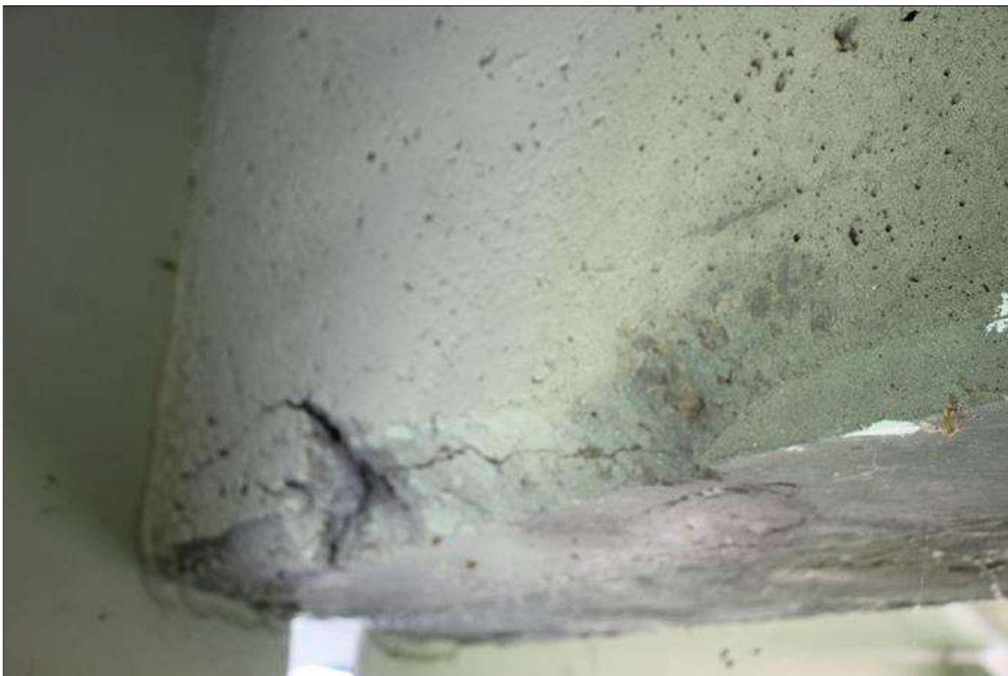
Span 2 Deck: UP TO 1.5 FT WIDE X 4 IN LONG X UP TO 2 IN DEEP SPALL IN DIAPHRAGM IN BAY 3 AT BENT 1.
