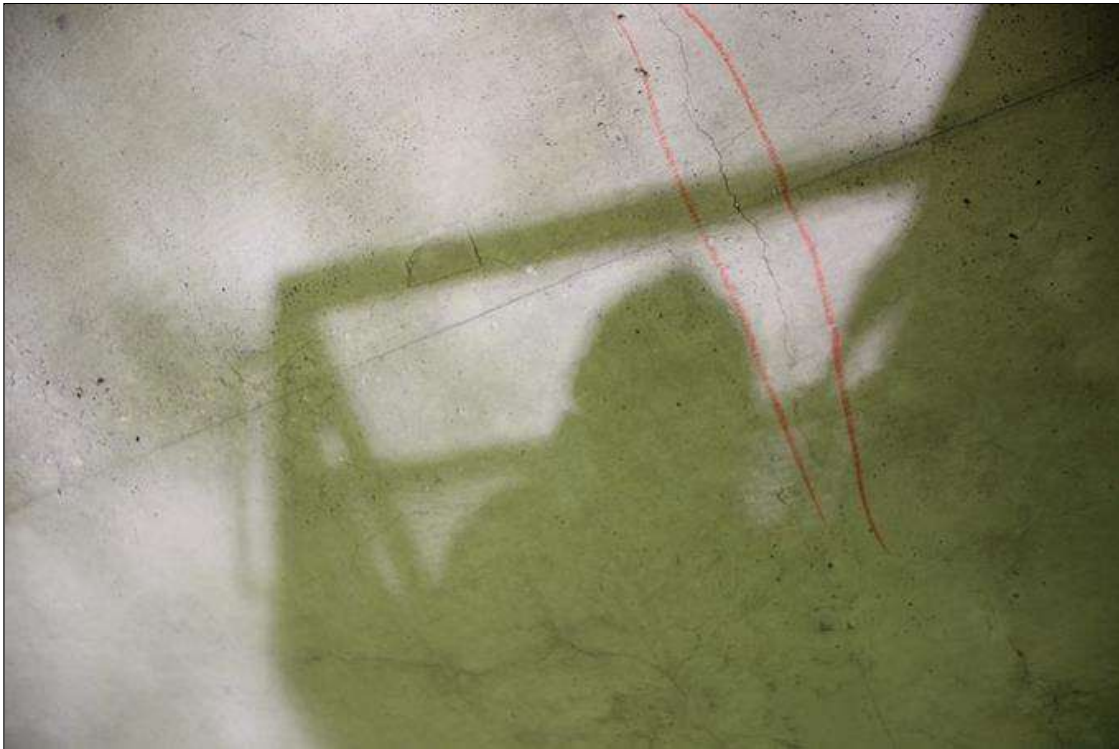
Span 3 Deck: UP TO 0.03 IN WIDE TRANSVERSE AND RANDOM CRACKING IN DECK UNDERSIDE IN ALL BAYS, SCATTERED THROUGHOUT. BAY 3 SHOWN IN PHOTO.
