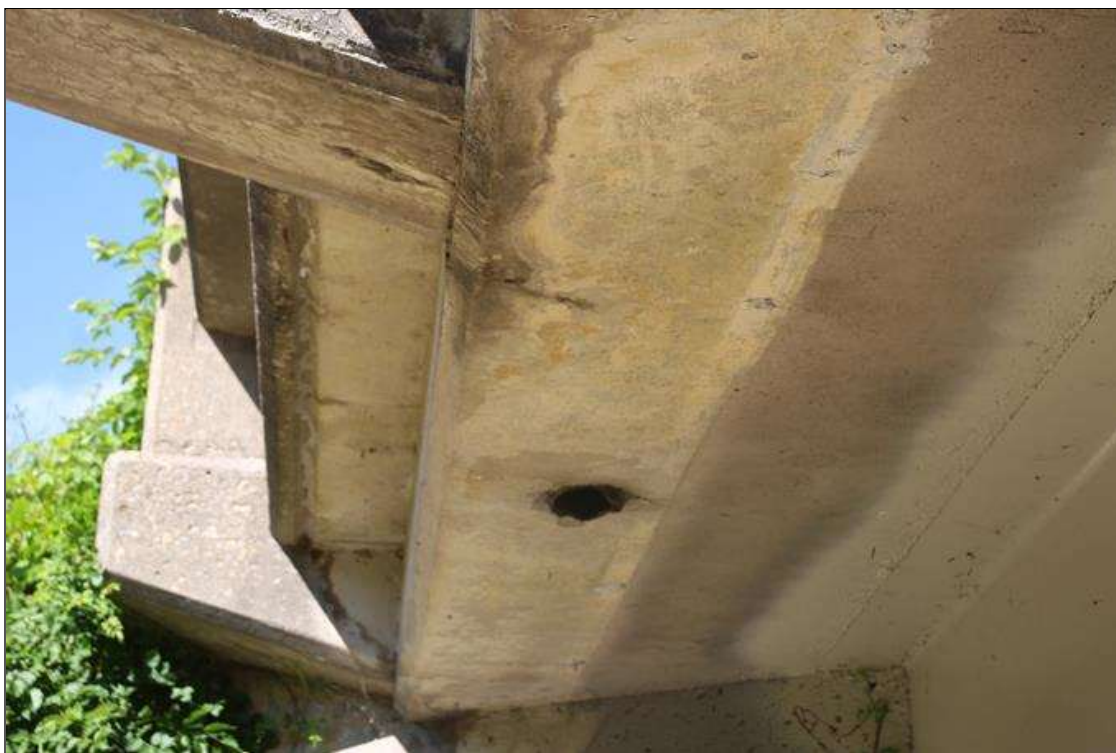
ONE BROKEN DRAIN PIPE AND THREE (3) PARTIALLY BROKEN DRAIN PIPES IN SPAN 1 RIGHT OVERHANG.
