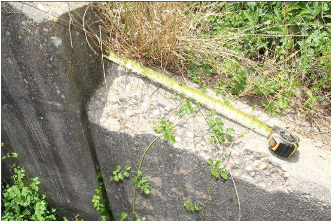
2 FT WIDE X 8 IN LONG X UP TO 5 IN DEEP SPALL IN THE TOP OF WINGWALL AT SOUTHWEST CORNER.
