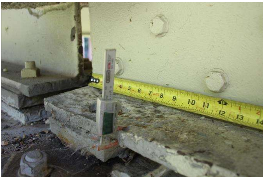
Span 2 Beam 1: 10 IN LONG X 5 IN WIDE AREA OF SECTION LOSS BENEATH THE PAINTED SURFACE ABOVE THE BEARING AT BENT 2. 0.60 IN SECTION REMAINING (PAR).
