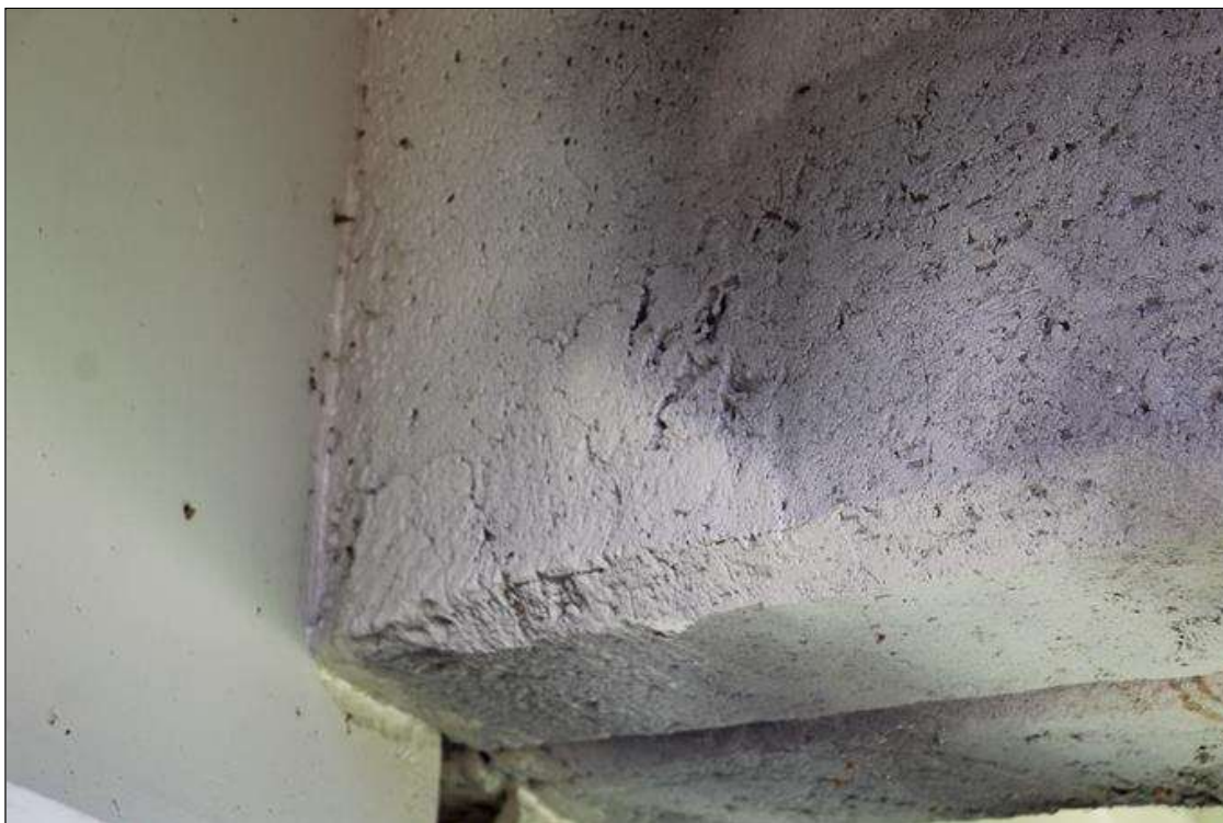
Span 7 Deck: NEW REPAIR: 2 FT HIGH X 1 FT WIDE SOUND CONCRETE PATCH IN DIAPHRAGM OUTSIDE BEAM 4 AT BENT 7.
