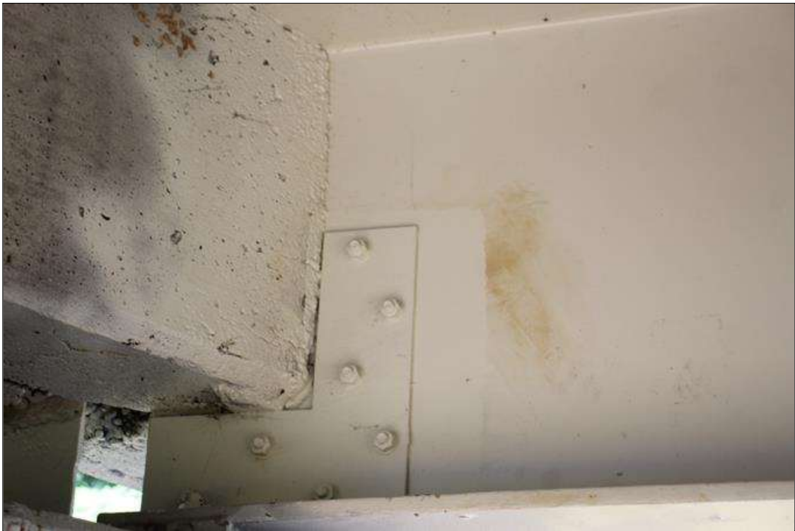
NEW REPAIR TO SPAN 5 BEAM 1 BEAM END IN BOTH FACES OF THE WEB ABOVE BENT 4.
