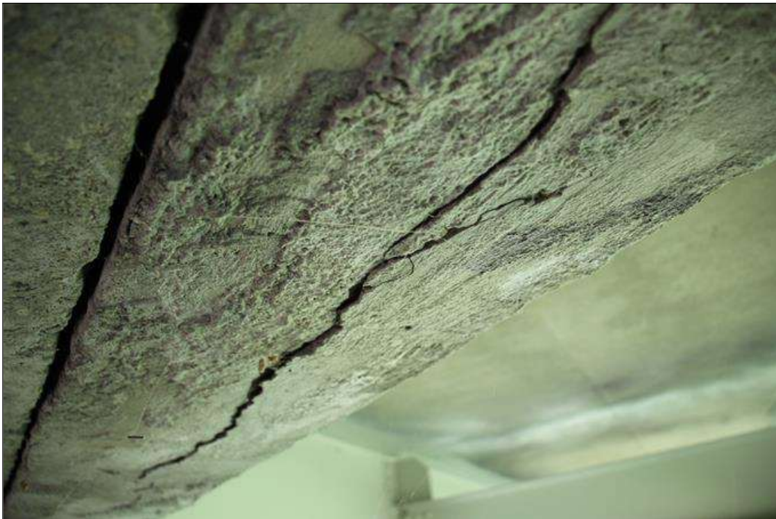
Span 2 Deck: 9 FT LONG X 1 FT HIGH SOUND CONCRETE PATCH, BAY 2 END DIAPHRAGM, AT BENT 2. PATCH EXHIBITS UP TO 1/8 IN WIDE X 5 FT LONG CRACK IN THE BOTTOM FACE WITH A 5 FT LONG X 5 IN WIDE UNSOUND CONCRETE AND UP TO 0.02 IN WIDE VERTICAL CRACKS IN FRON FACE, SCATTERED.
