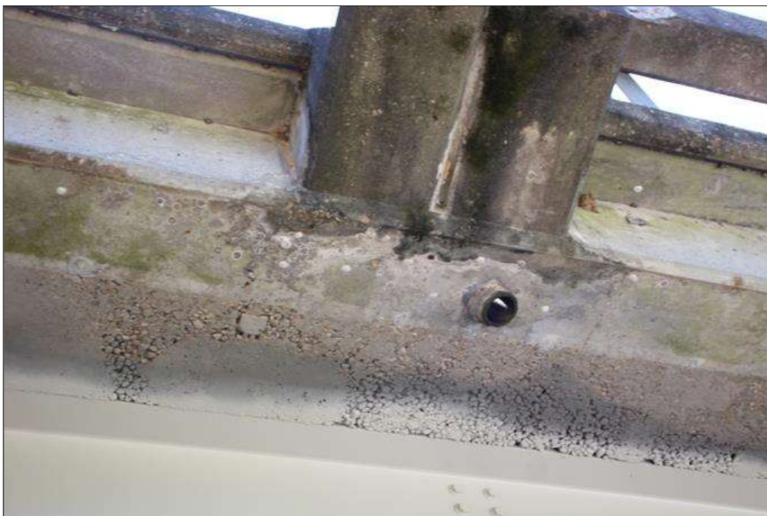
Span 4 Deck: 7 FT LONG X 2 FT LONG AREA OF HONEYCOMBING LOCATED AT MID SPAN.
