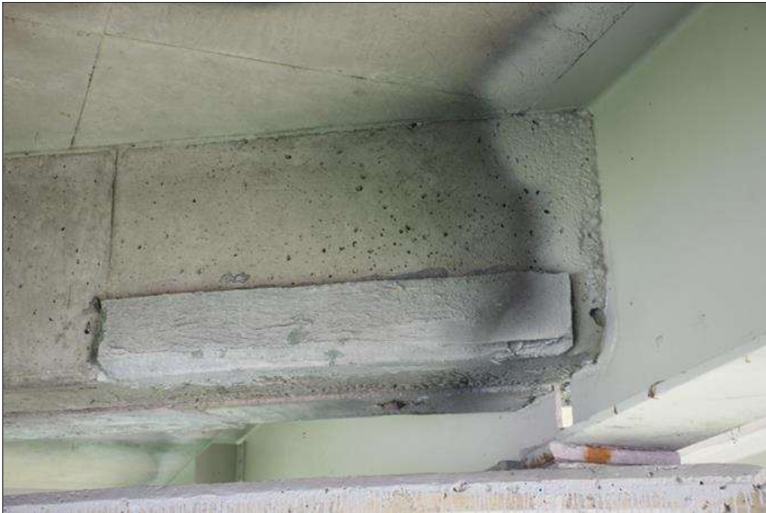
Span 1 Deck: 4 FT LONG X 8 IN HIGH SOUND CONCRETE PATCH IN BAY 2 END DIAPHRAGM, AT BENT 1.
