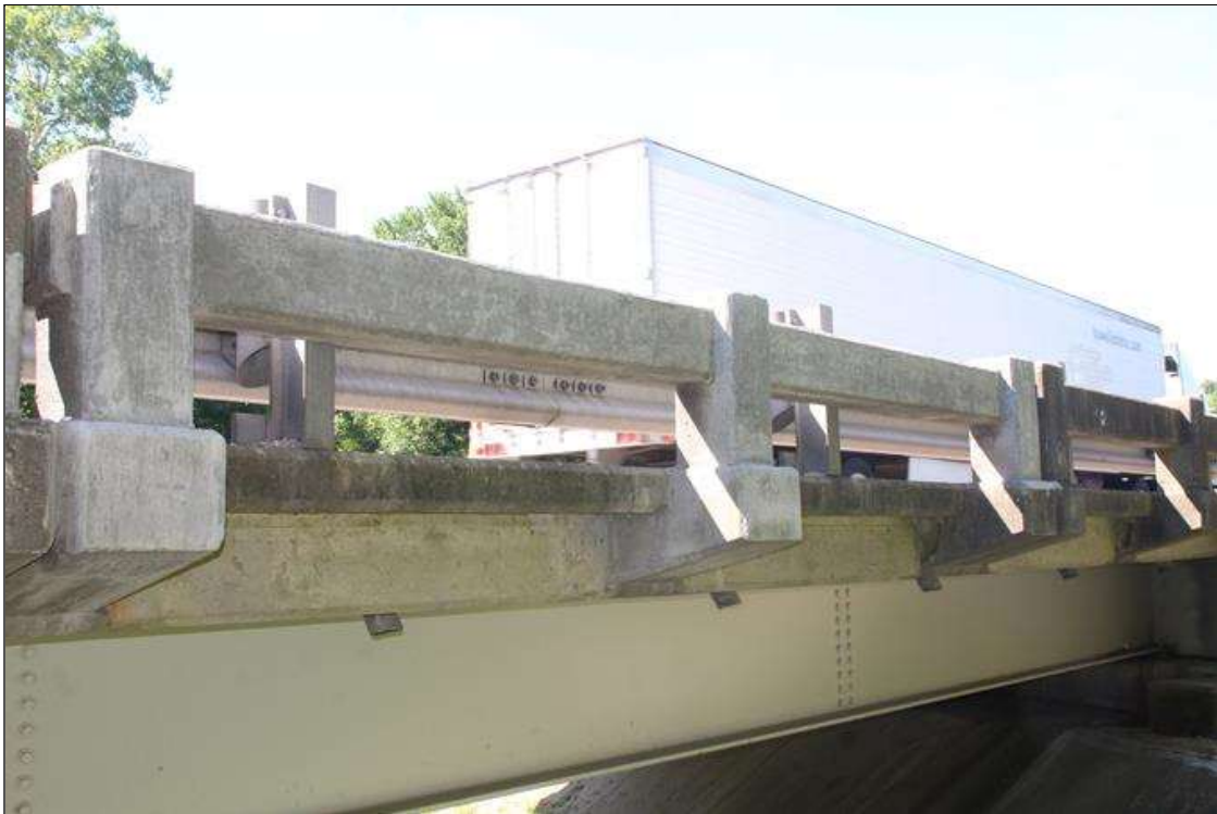
Span 1 Left Bridge Rail: 15 FT LONG AREA OF SOUND CONCRETE PATCHING TO CONCRETE RAIL, BEGINNING AT 15 FT FROM END BENT 1. PREVIOUS REPAIR.
