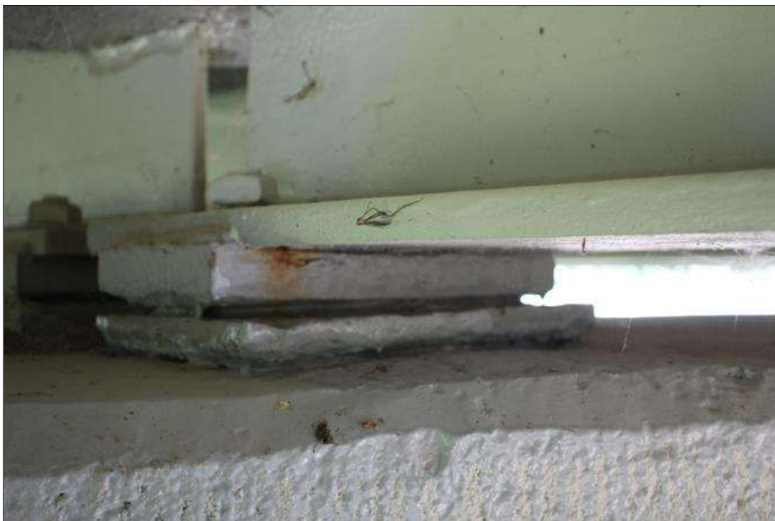
Span 7 Beam 2 Far Bearing: BEARINGS HAVE BEEN PAINTED SINCE PREVIOUS INSPECTION. SECTION LOSS REMAINS BENEATH THE PAINTED SURFACES. UP TO 80% SECTION REMAINING IN BOTH MASONRY AND SOLE PLATES.
