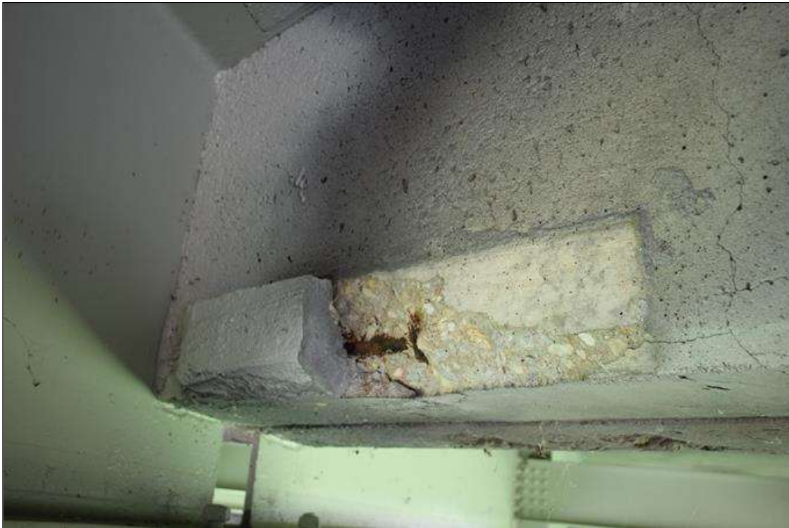
Span 3 Deck: 3 FT LONG X 6 IN HIGH UNSOUND CONCRETE PATCH WITH EXPOSED REINFORCEMENT. 90% SECTION REMAINING IN EXPOSED REINFORCEMENT.
