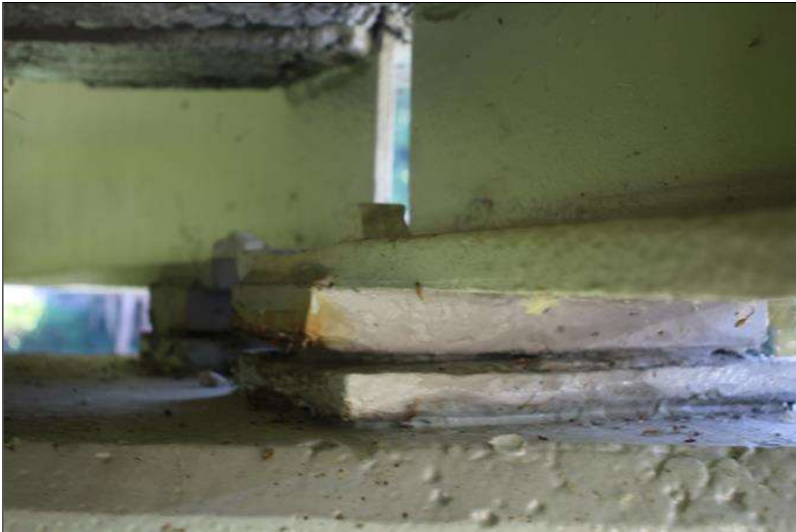
Span 1 Beam 4 Far Bearing: SECTION LOSS IN THE RIGHT ANCHOR BOLT. 75% SECTION REMAINING.
