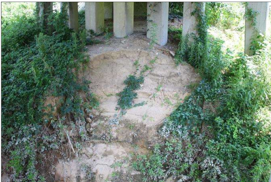
20 FT WIDE X 50 FT LONG X UP TO 5 FT HIGH AREA OF EROSION IN THE SLOPE UNDER SPAN 7.
