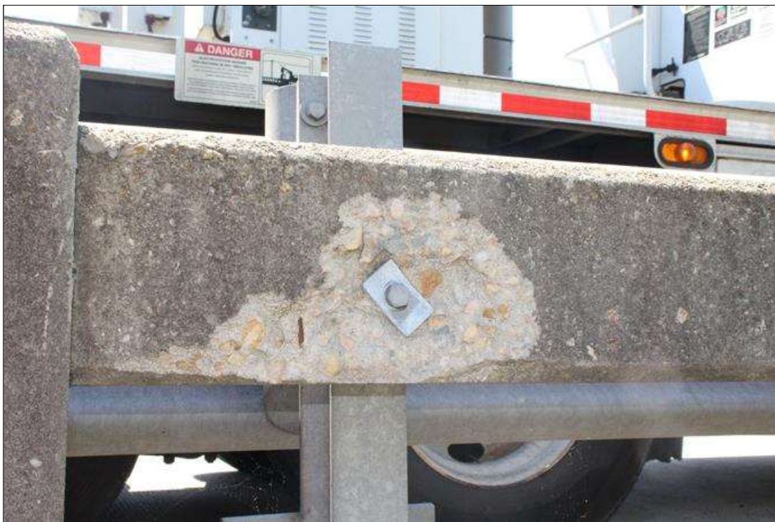
Span 4 Right Bridge Rail: 1.5 FT LONG X 9 IN HIGH X UP TP 1.5 IN DEEP SPALL IN EXTERIOR FACE OF RAIL, LOCATED AT MID SPAN.
