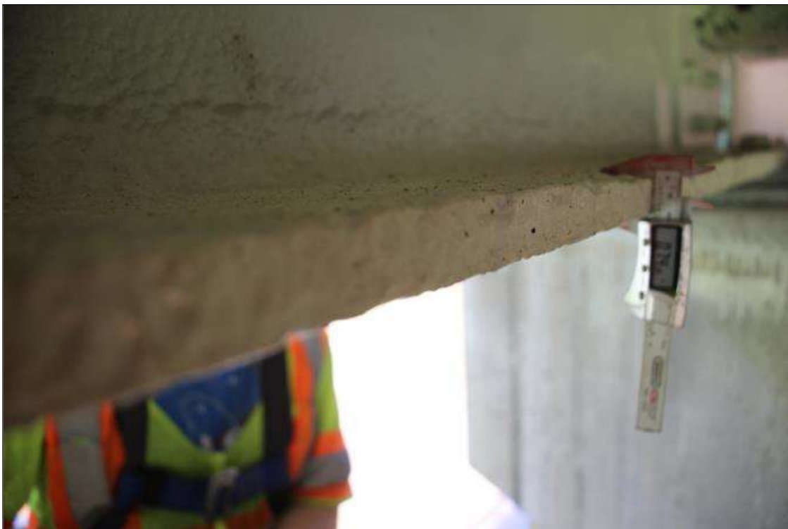
Span 3 Beam 1: 2 FT LONG X 5 IN WIDE AREA OF BOTTOM FLANGE HAS SECTION LOSS BENEATH THE PAINTED SURFACE, LOCATED AT 2 FT FROM BEAM END AT BENT 3. 0.74 IN SECTION REMAINING.
