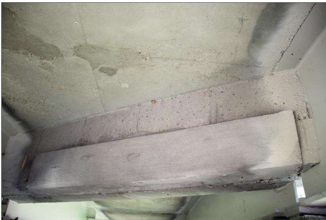
Span 7 Deck: 7 FT LONG X 1 FT HIGH SOUND CONCRETE PATCH IN INTERMEDIATE DIAPHRAGM IN BAY 3 AT BENT 7.
