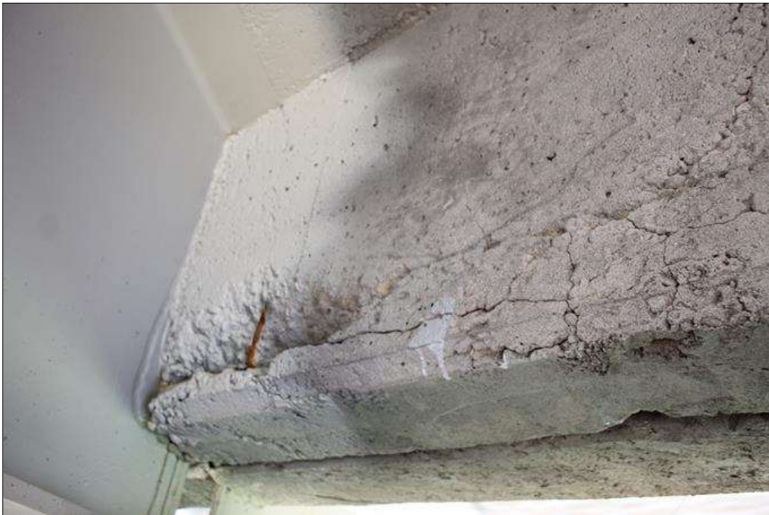
Span 6 Deck: 2.5 FT WIDE X 10 IN LONG X UP TO 6 IN HIGH AREA OF UNSOUND CONCRETE AND SPALL UP TO 2 IN DEEP WITH EXPOSED REINFORCEMENT IN BAY 3 END DIAPHRAGM AT BENT 7. NO MEASUREABLE SECTION LOSS IN EXPOSED REINFORCEMENT.
