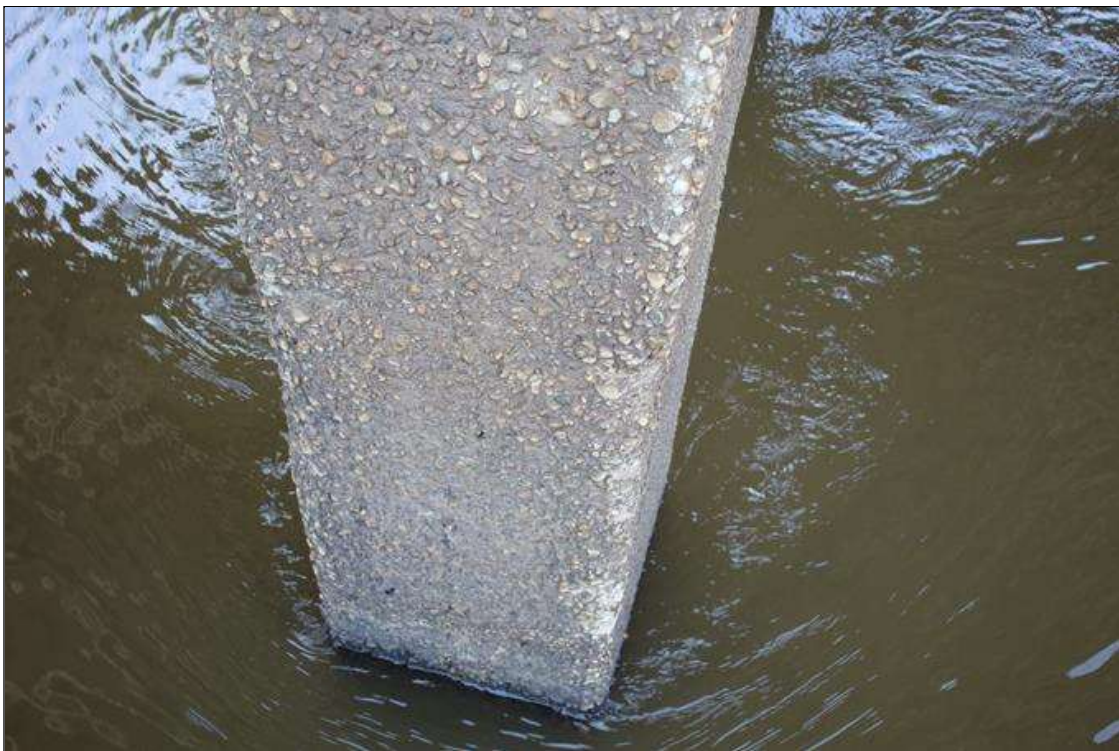
Bent 5 Pile 1: ABRASION WITH COARSE AGGREGATE EXPOSED 1/16 IN TO 1/4 IN LOSS OF FACIAL CONCRETE.
