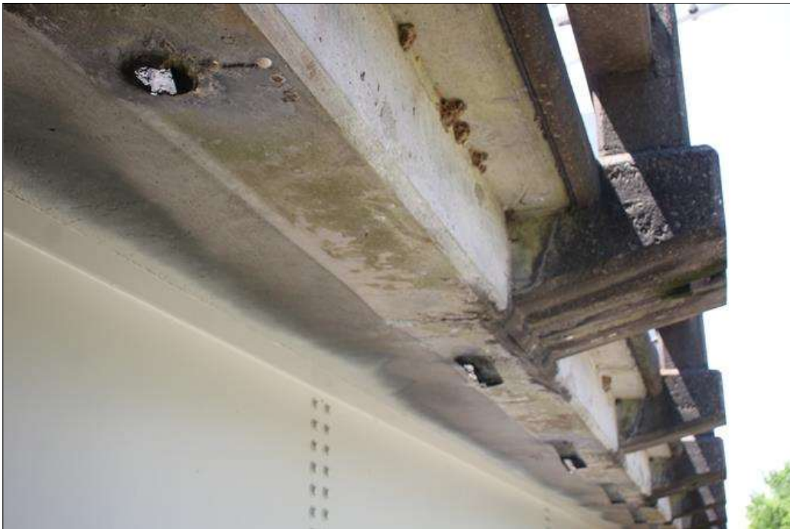
DECK DRAINS ALONG LEFT BRIDGE RAIL IN SPAN 6. ONE DRAIN BROKEN OFF AND TWO (2) PARTIALLY BROKEN.
