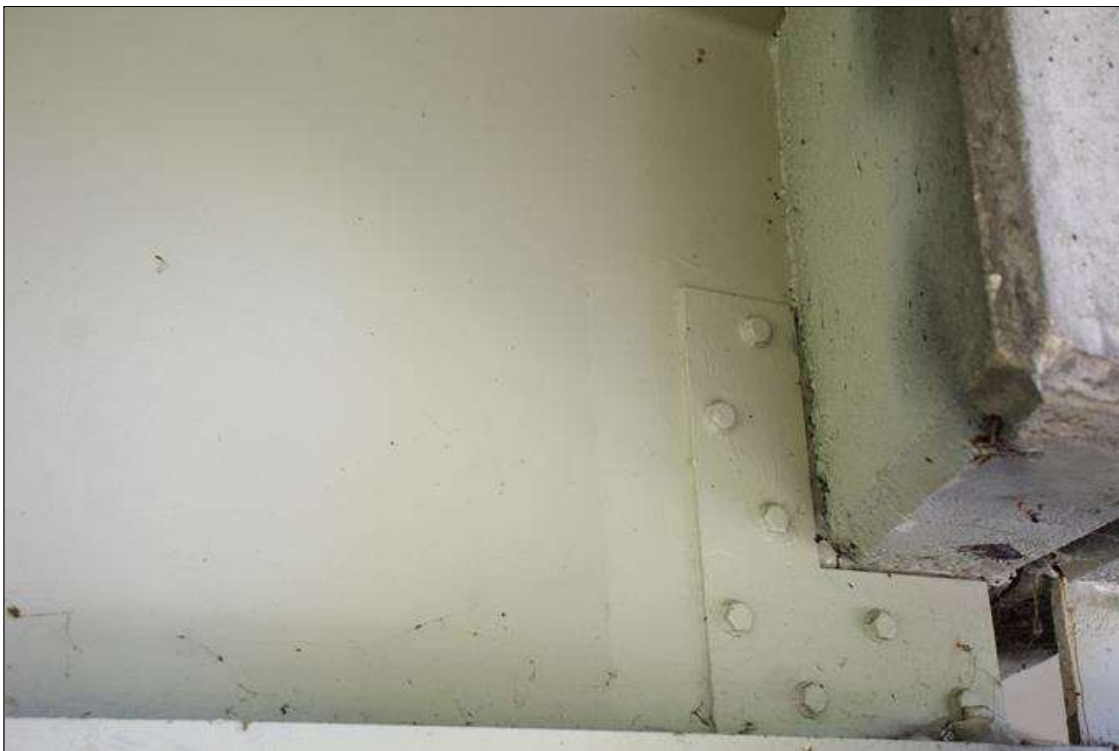
NEW REPAIR TO SPAN 8 BEAM 1 BEAM END IN BOTH FACES OF THE WEB ABOVE BENT 7.
