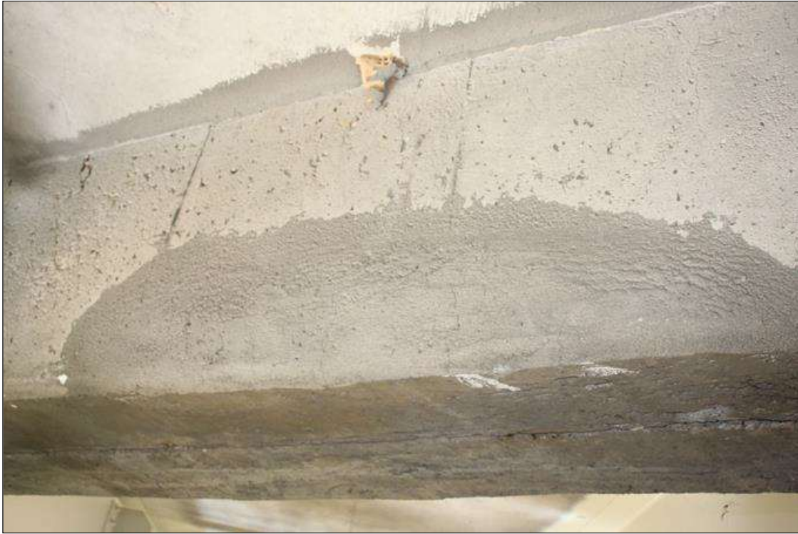
Span 6 Deck: NEW REPAIR: 28 IN LONG X 1 FT HIGH SOUND CONCRETE PATCH IN BAY 2 END DIAPHRAGM, AT BENT 5. PATCH EXHIBITS HAIRLINE VERTICAL CRACKING, SCATTERED.
