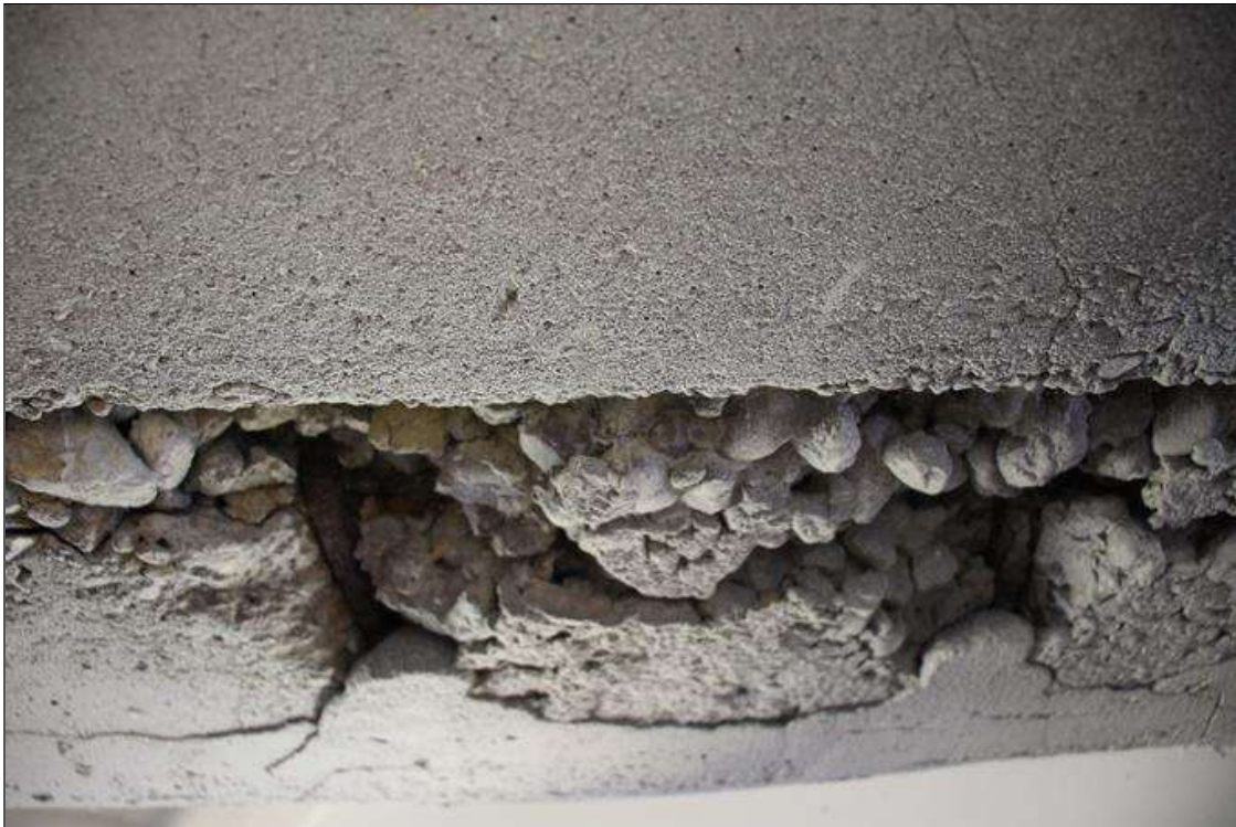
Span 4 Deck: 2 IN WIDE X 7 IN LONG X UP TO 2 IN DEEP SPALLS AND HONEYCOMBING WITH EXPOSED REBAR IN BOTTOM OF DIAPHRAGM IN BAY 1 AT BENT 4. NO MEASUREABLE SECTION LOSS IN EXPOSED REINFORCEMENT.
