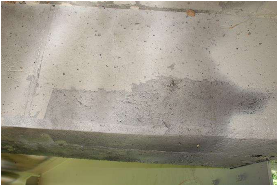
Span 4 Deck: 2.5 FT LONG X 6 IN HIGH SOUND CONCRETE PATCH WITH HAIRLINE VERTICAL CRACKS IN BAY 1 ABOVE BENT 3.
