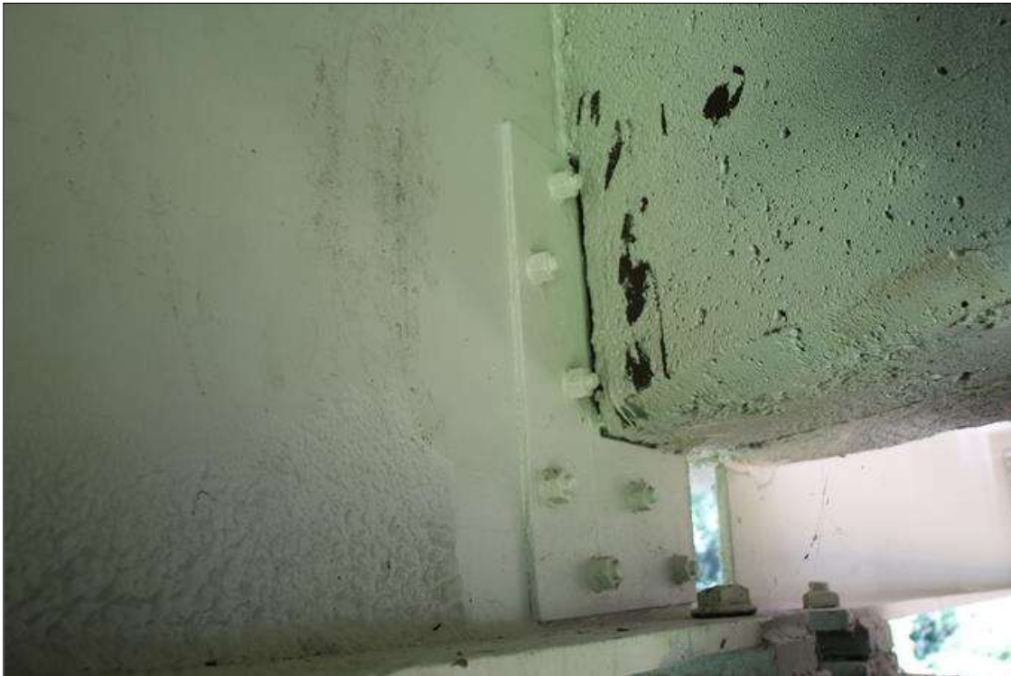
NEW REPAIR TO SPAN 3 BEAM 1 BEAM END IN BOTH FACES OF THE WEB ABOVE BENT 3.
