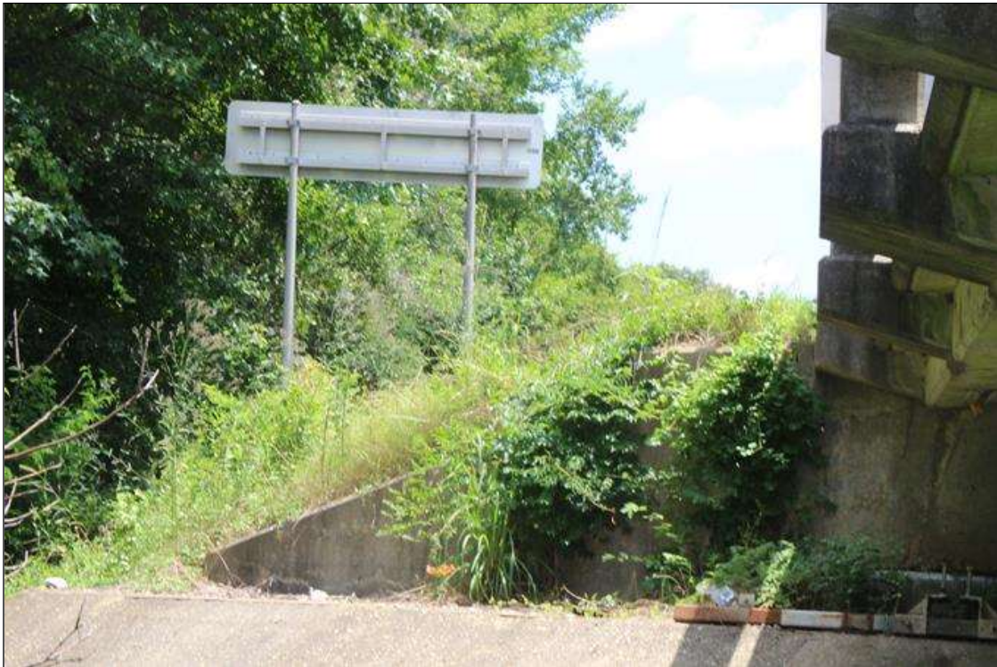
NORTHWEST WINGWALL. NOTE HEAVY VEGETATION GROWTH.
