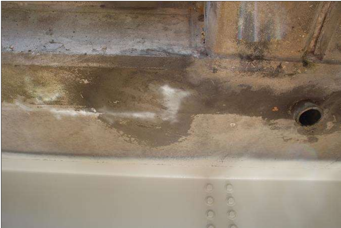
Span 6 Deck: NEW REPAIR: 18 IN DIAMETERE SOUND CONCRETE PATCH IN EAST OVERHANG BETWEEN 5TH AND 6TH DECK DRAINS.
