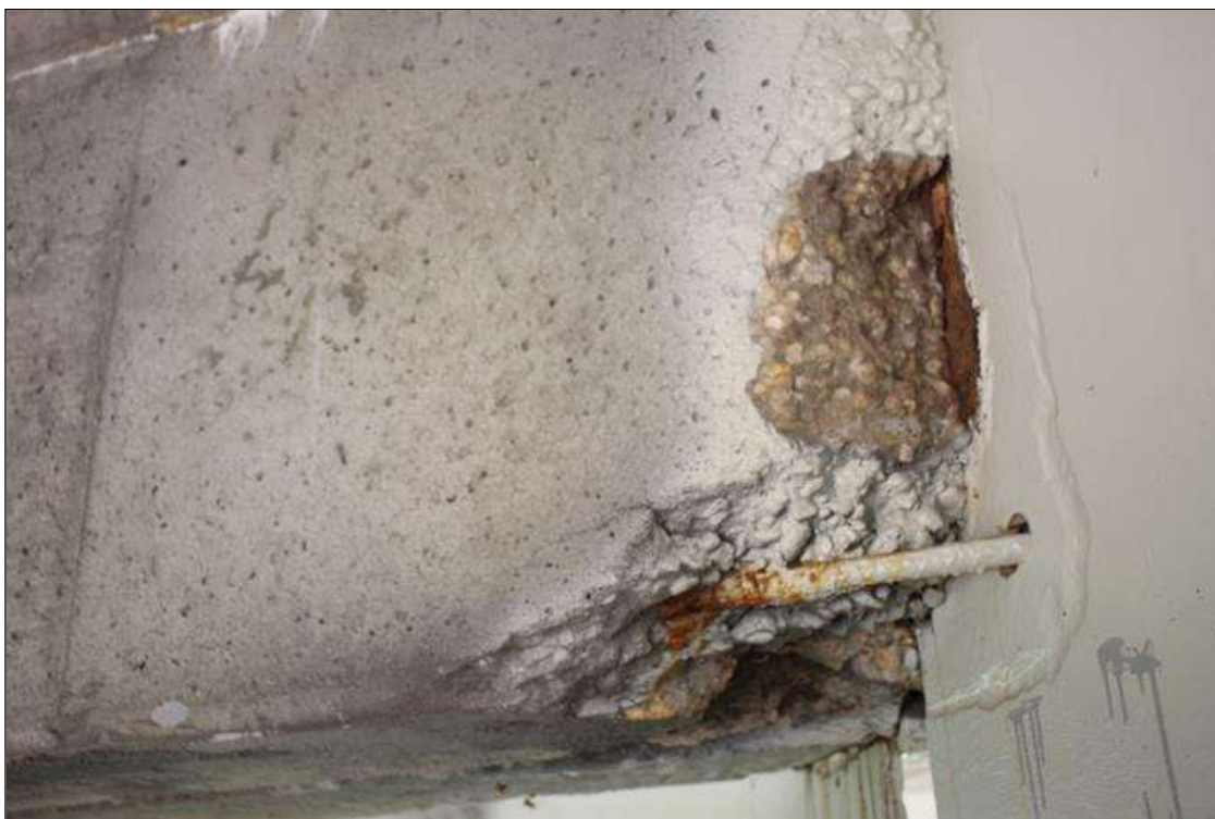
Span 6 Deck: 12 IN WIDE X 9 IN LONG X 14 IN HIGH IN SOUTH FACE SPALL UP TO 3.5 IN DEEP WITH EXPOSED REINFORCEMENT IN BAY 2 AT BENT 6. NO MEASUREABLE SECTION LOSS IN EXPOSED REINFORCEMENT.
