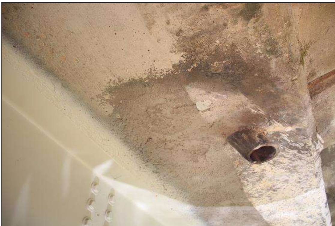
Span 7 Deck: NEW REPAIR: 18 IN DIAMETER SOUND CONCRETE PATCH IN EAST OVERHANG AT THIRD DRAIN PIPE.
