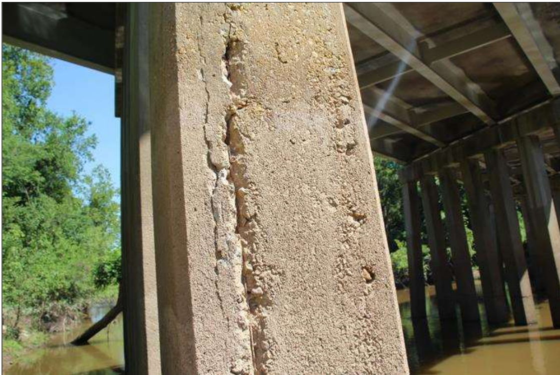
Bent 3 Pile 7: 4 FT HIGH X 4 IN WIDE SPALL WITH EXPOSED REINFORCEMENT IN EAST FACE. 90% SECTION REMAINING IN EXPOSED REINFORCEMENT (PAR).
