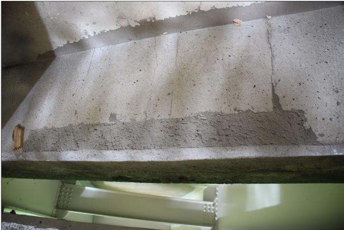
Span 4 Deck: 4 FT LONG X 6 IN HIGH SOUND CONCRETE PATCH WITH HAIRLINE VERTICAL CRACKS IN BAY 2 AT BENT 3.
