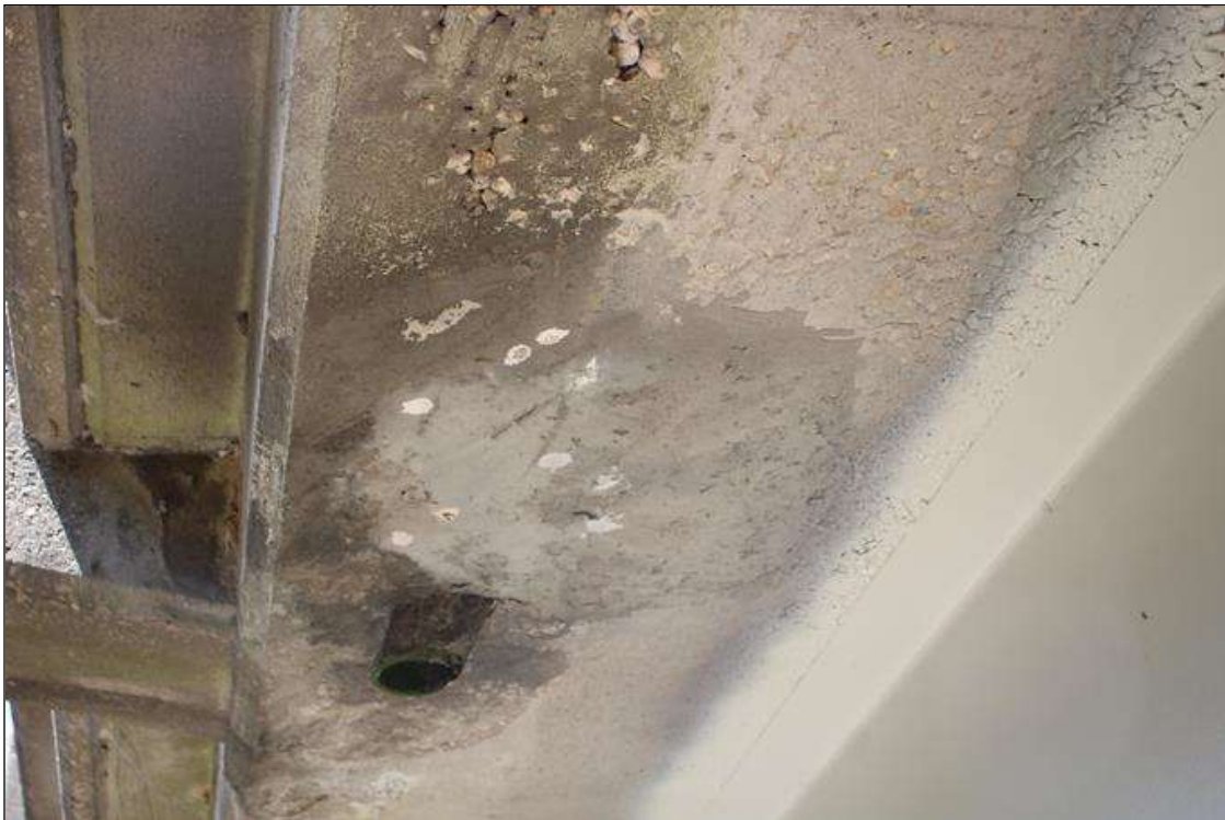
Span 6 Deck: NEW REPAIR: 12 IN DIAMETER SOUND CONCRETE PATCH IN EAST OVERHANG AT DRAIN ONE.
