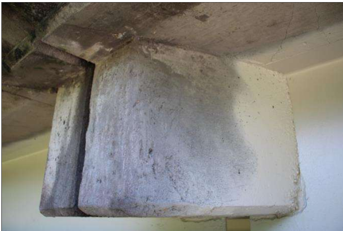
Span 6 Deck: NEW REPAIR: 2 FT HIGH X 1 FT WIDE SOUND CONCRETE PATCH IN END DIAPHRAGM OUTSIDE BEAM 1 AT BEAM 6.
