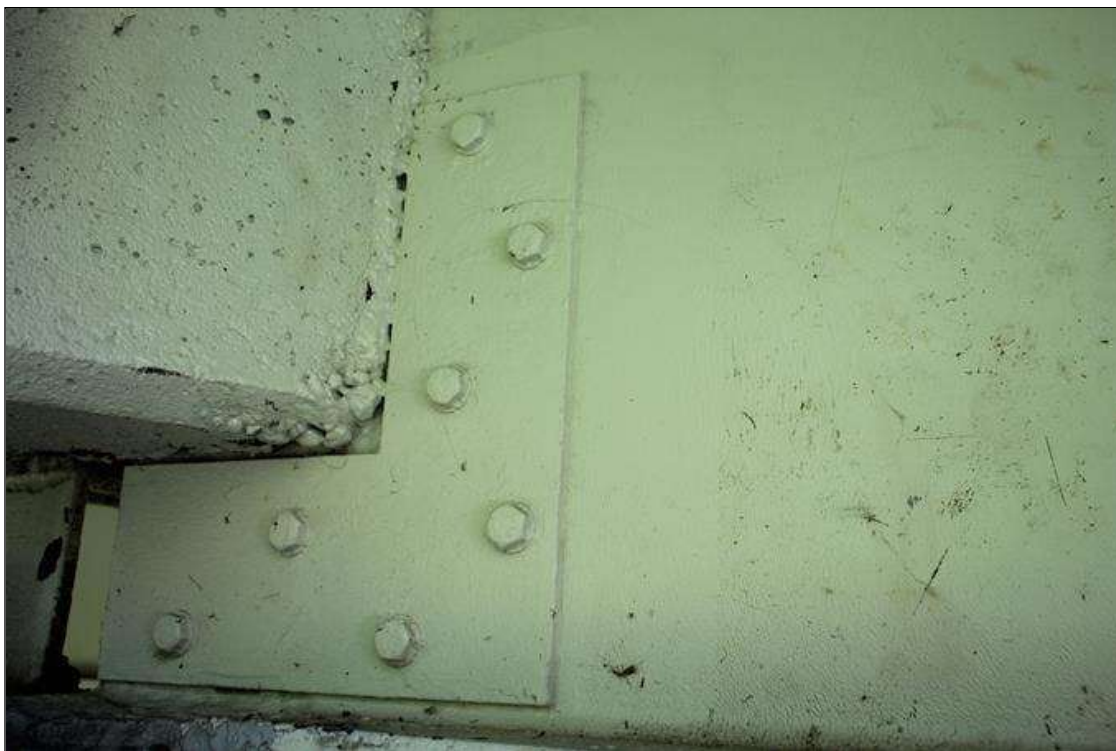
NEW REPAIR TO SPAN 2 BEAM 1 BEAM END IN BOTH FACES OF THE WEB ABOVE BENT 2.
