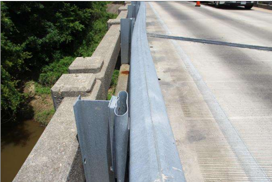
Span 6 Left Bridge Rail: MODERATE TO HEAVY IMPACT DAMAGE WITH UP TO 5 IN DEFLECTION TOWARDS WEST TO THE SUPPLEMENTAL BRIDGE RAIL FOR 20 FT LONG STARTING AT BENT 6. TWO (2) SPACER BLOCKS CONNECTING THE GUARDRAIL TO POSTS ARE PARTIALLY CRUSHED.
