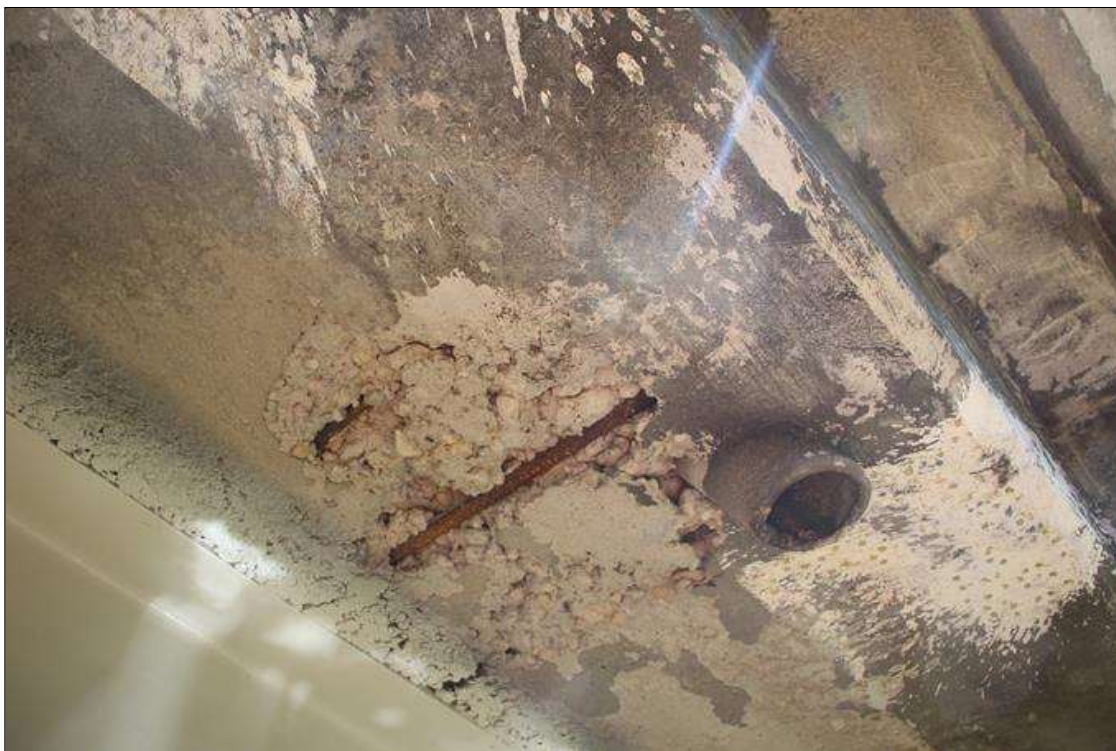
Span 7 Deck: 24 IN LONG X 2 FT WIDE X 2 IN DEEP DELAMINATION/SPALL WITH EXPOSED REINFORCING, UNDERSIDE OF EAST OVERHANG AT 2/3 POINT. NO MEASUREABLE SECTION LOSS IN EXPOSED REINFORCEMENT.
