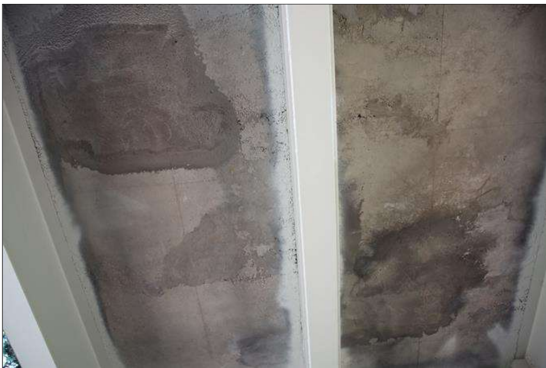
Span 7 Deck: 75 SQ FT OF PATCHED AREA, UNDERSIDE OF DECK, AT RANDOM THROUGHOUT ALL BAYS. PHOTO SHOWS BAYS 1 AND 2.
