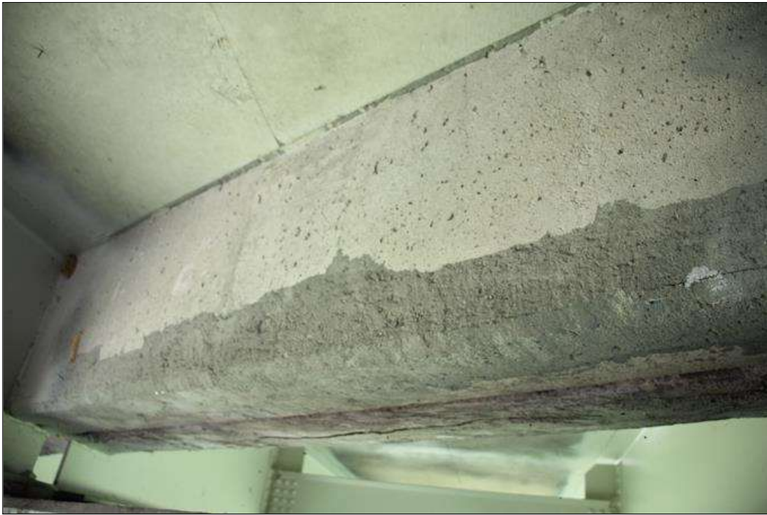
Span 3 Deck: 7 FT LONG X 6 IN HIGH SOUND CONCRETE PATCH IN BAY 2 END DIAPHRAGM, AT BENT 2.
