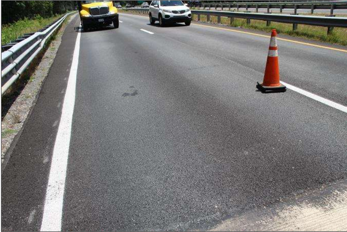
NEW APPROACH PAVEMENT IN NORTH APPROACH. TYPICAL IN SOUTH APPROACH.
