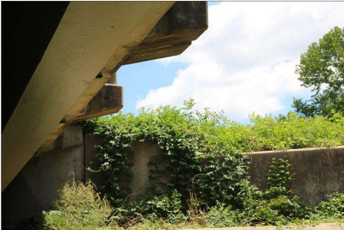
NORTHEAST WINGWALL. NOTE HEAVY VEGETATION.
