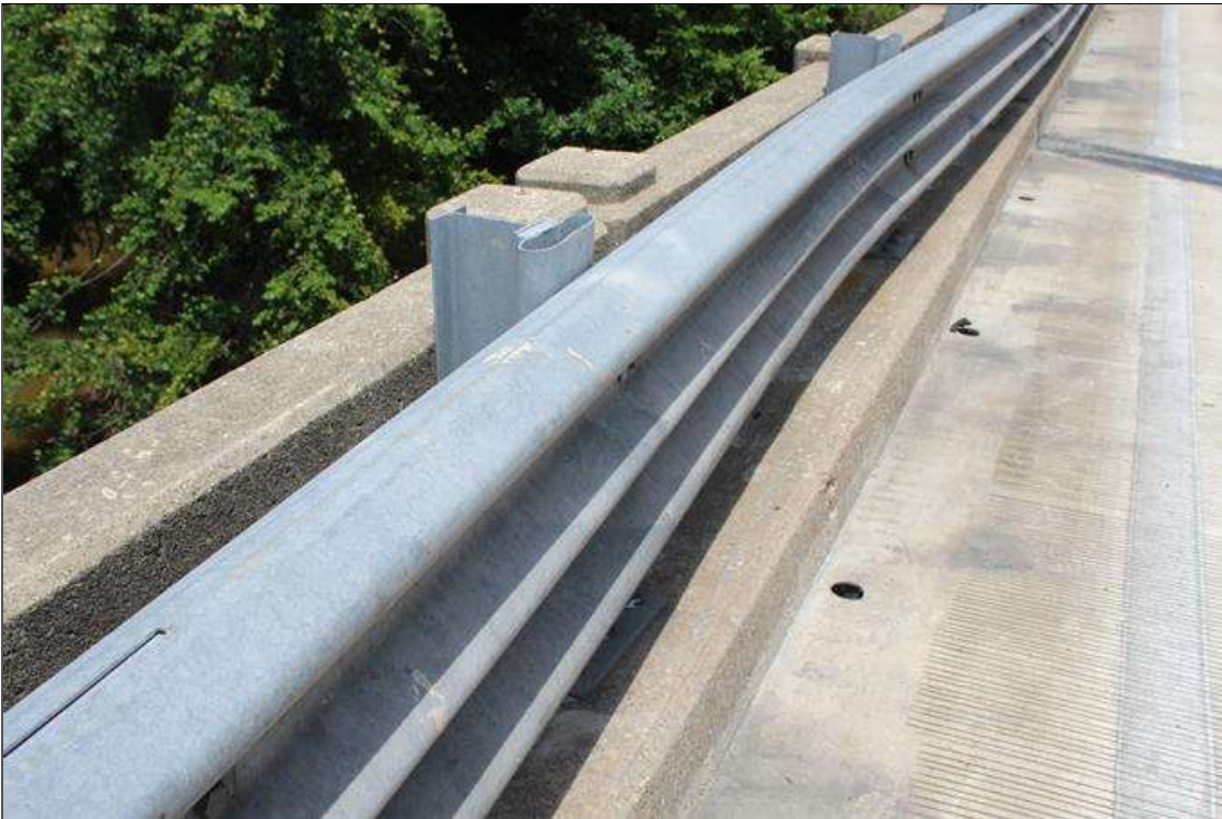
Span 6 Left Bridge Rail: MODERATE TO HEAVY IMPACT DAMAGE WITH UP TO 5 IN DEFLECTION TOWARDS WEST TO THE SUPPLEMENTAL BRIDGE RAIL FOR 20 FT LONG STARTING AT BENT 6. TWO (2) SPACER BLOCKS CONNECTING THE GUARDRAIL TO POSTS ARE PARTIALLY CRUSHED.
