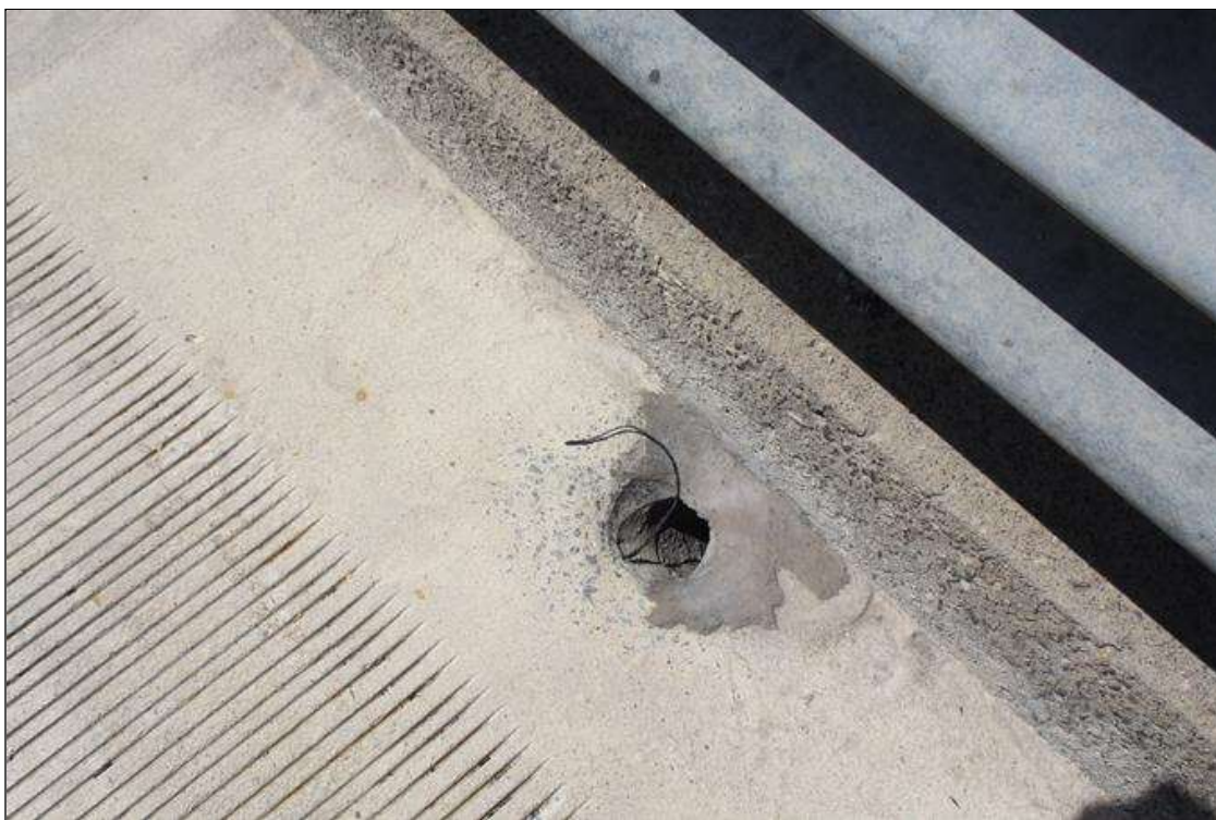
DECK DRAINS ALONG LEFT BRIDGE RAIL IN SPAN 8. TYPICAL ALONG BOTH BRIDGE RAILS AND IN ALL SPANS.
