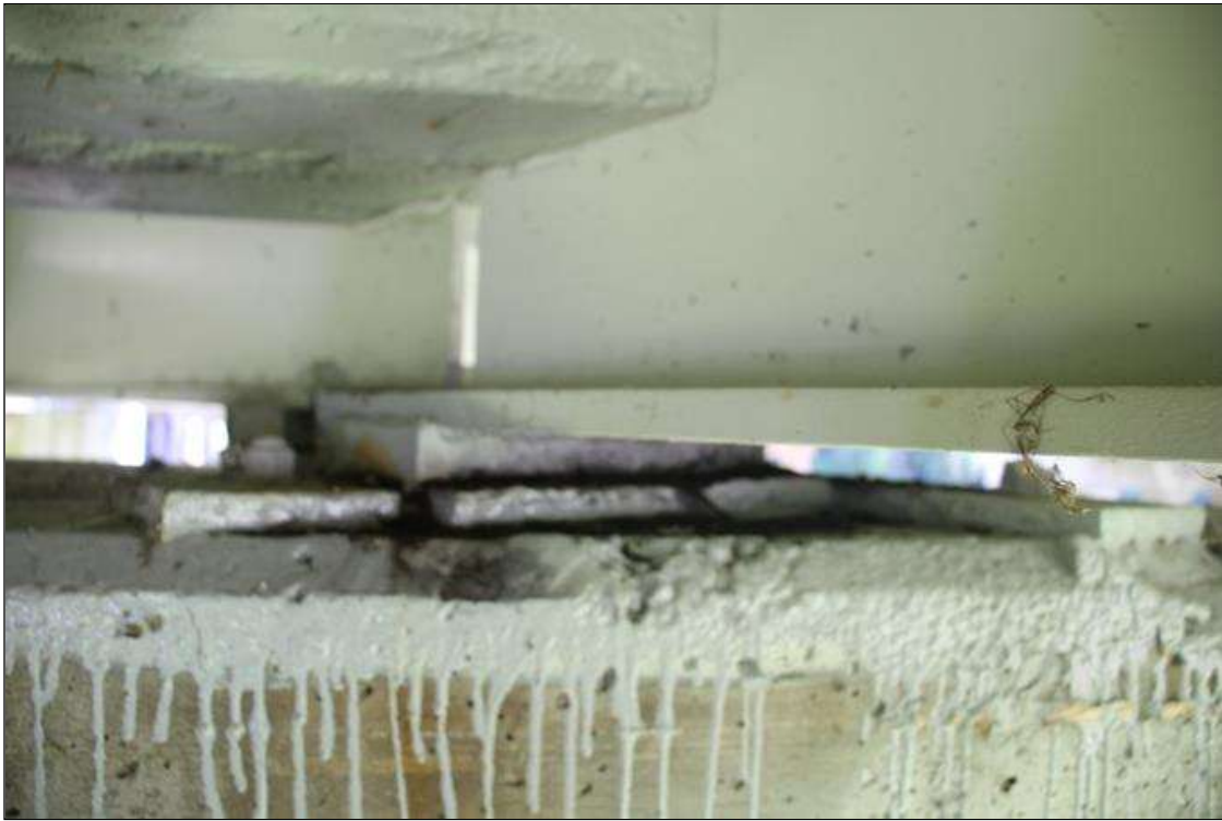
Span 2 Beam 3 Far Bearing: WELDED BEARING REPAIR WITH ANCHOR ROD. TYPICAL AT BEAMS 1, 2, AND 4.
