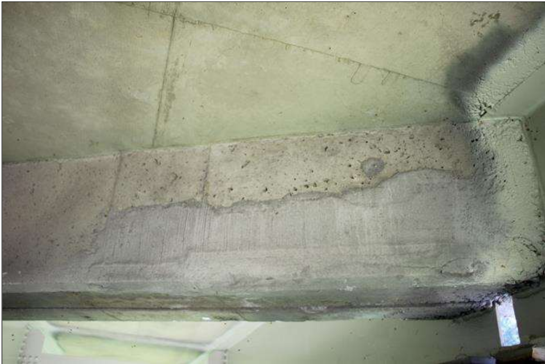
Span 1 Deck: 5 FT WIDE X 1 FT HIGH SOUND CONCRETE PATCH IN BAY 3 END DIAPHRAGM, AT BENT 1. PATCH EXHIBITS A HAIRLINE X 1 FT LONG CRACK IN BOTTOM RIGHT CORNER.
