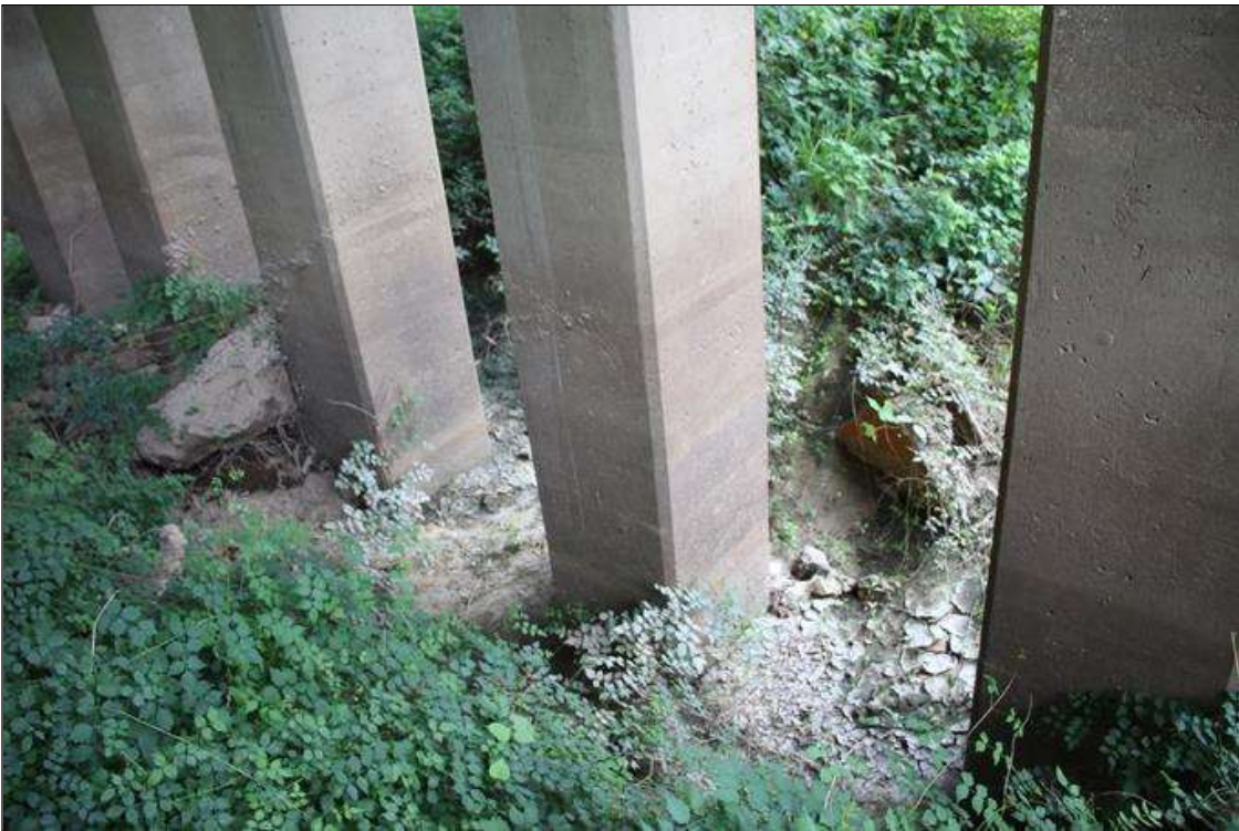
UP TO 2 FT OF EROSION ALONG THE PILES AT BENT 1.
