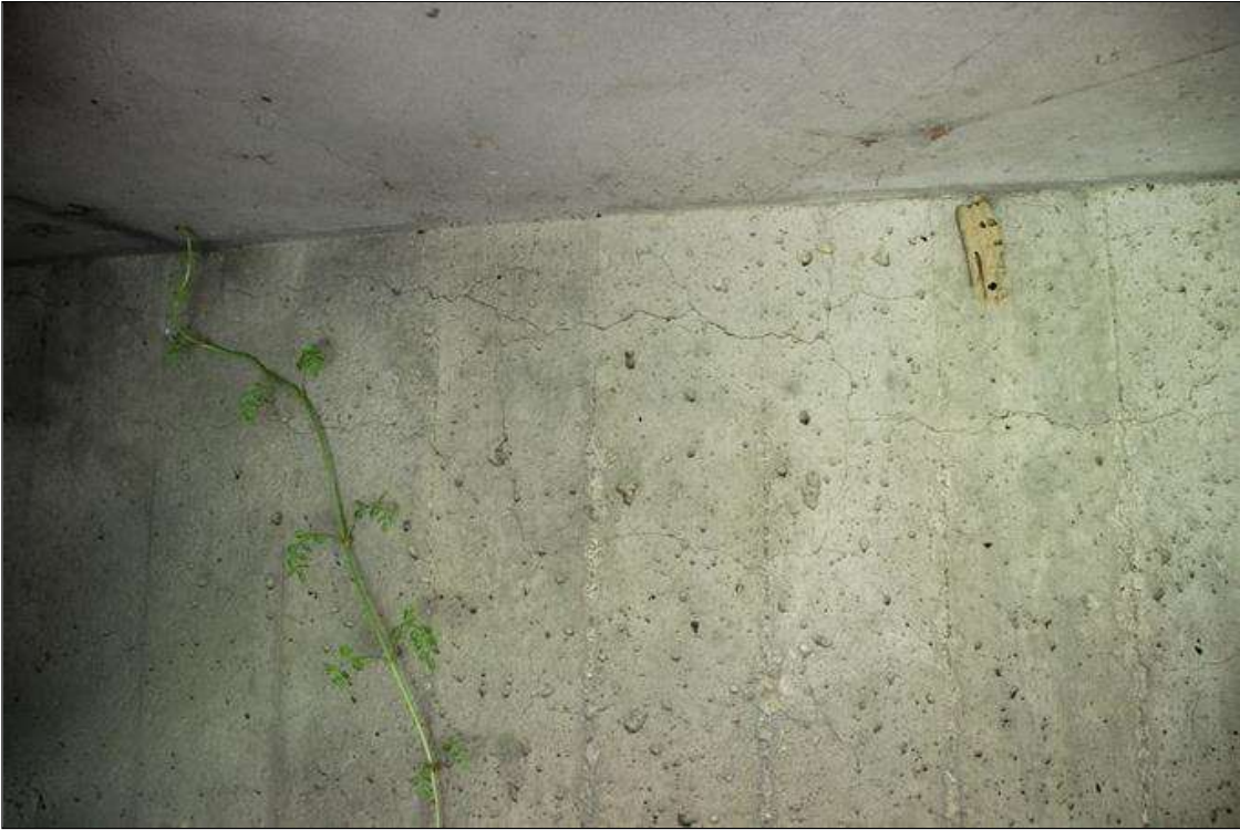
End Bent 1 Abutment/Backwall : UP TO 0.03 IN WIDE RANDOM CRACKING IN BACKWALL FOR FULL LENGTH.
