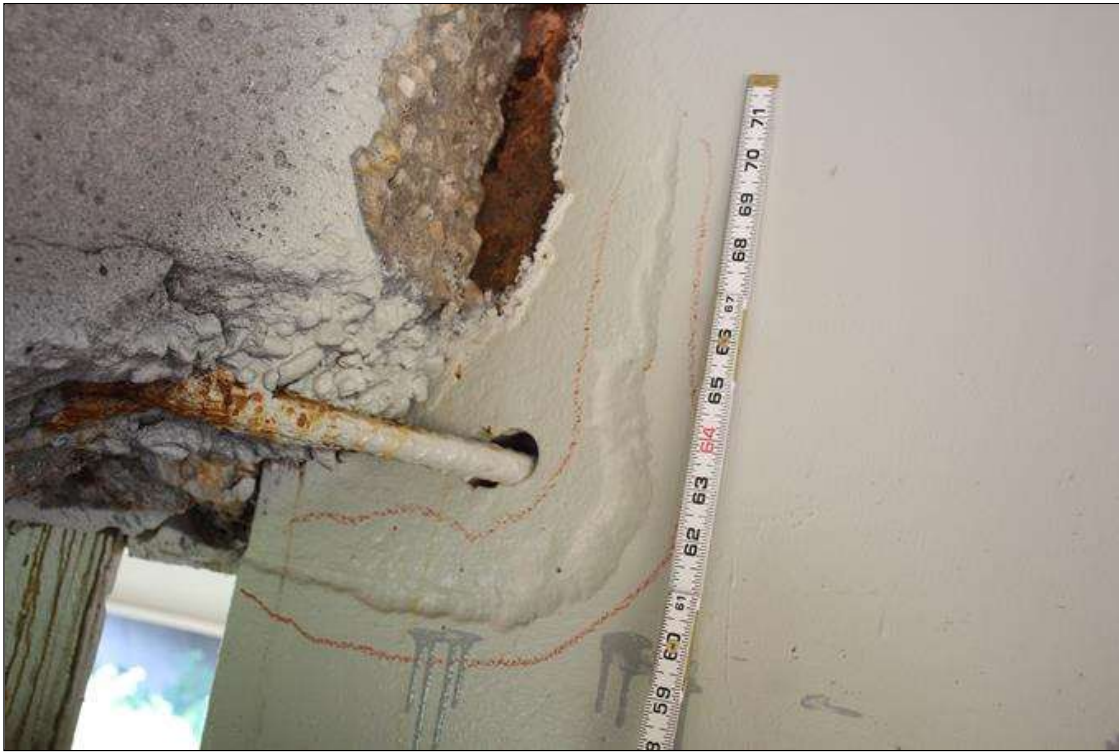
Span 6 Beam 3: UP TO 11 IN HIGH X 10 IN LONG AREA OF SECTION LOSS IN THE WEB BENEATH THE PAINTED SURFACE AT BEAM END AT BENT 6. 0.575 IN SECTION REMAINING.
