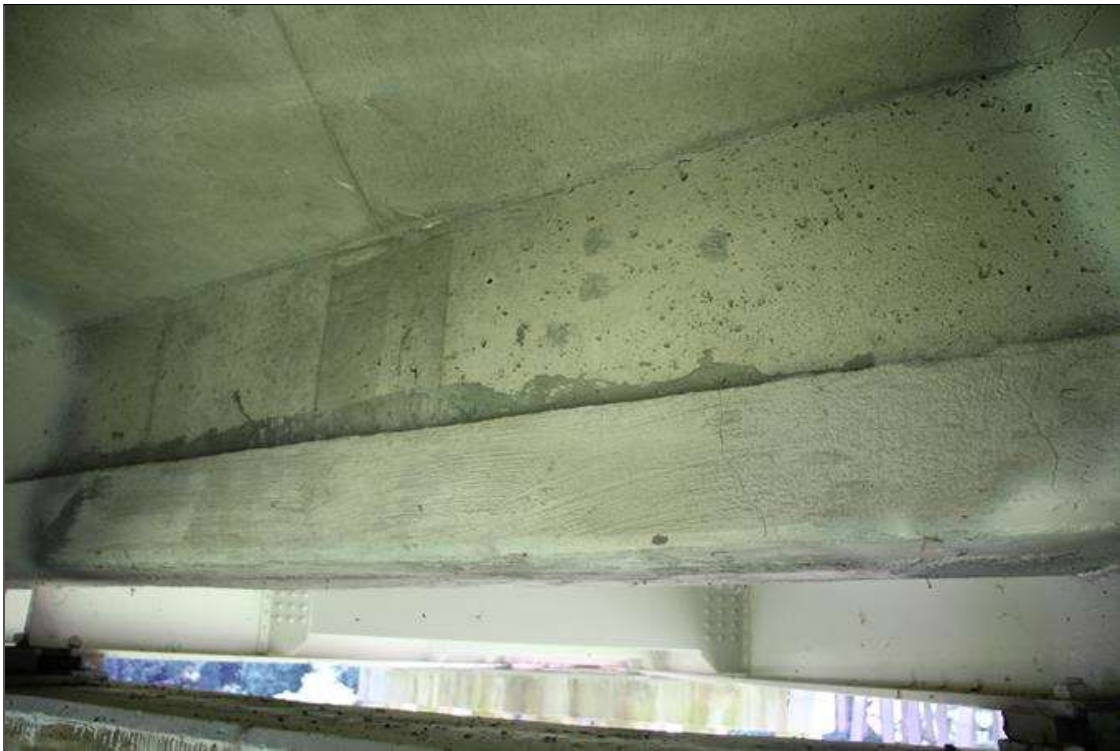
Span 2 Deck: 9 FT LONG X 1 FT HIGH CONCRETE PATCH, BAY 2 END DIAPHRAGM, AT BENT 2. PATCH EXHIBITS UP TO 1/8 IN WIDE X 5 FT LONG CRACK IN THE BOTTOM FACE WITH A 5 FT LONG X 5 IN WIDE UNSOUND CONCRETE AND UP TO 0.02 IN WIDE VERTICAL CRACKS IN FRONT FACE, SCATTERED.
