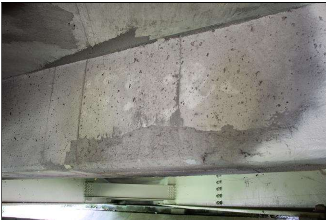
Span 7 Deck: NEW REPAIR 2 FT HIGH X 1 FT WIDE SOUND CONCRETE PATCH IN DIAPHRAGM OUTSIDE BEAM 4 AT BENT 7.
