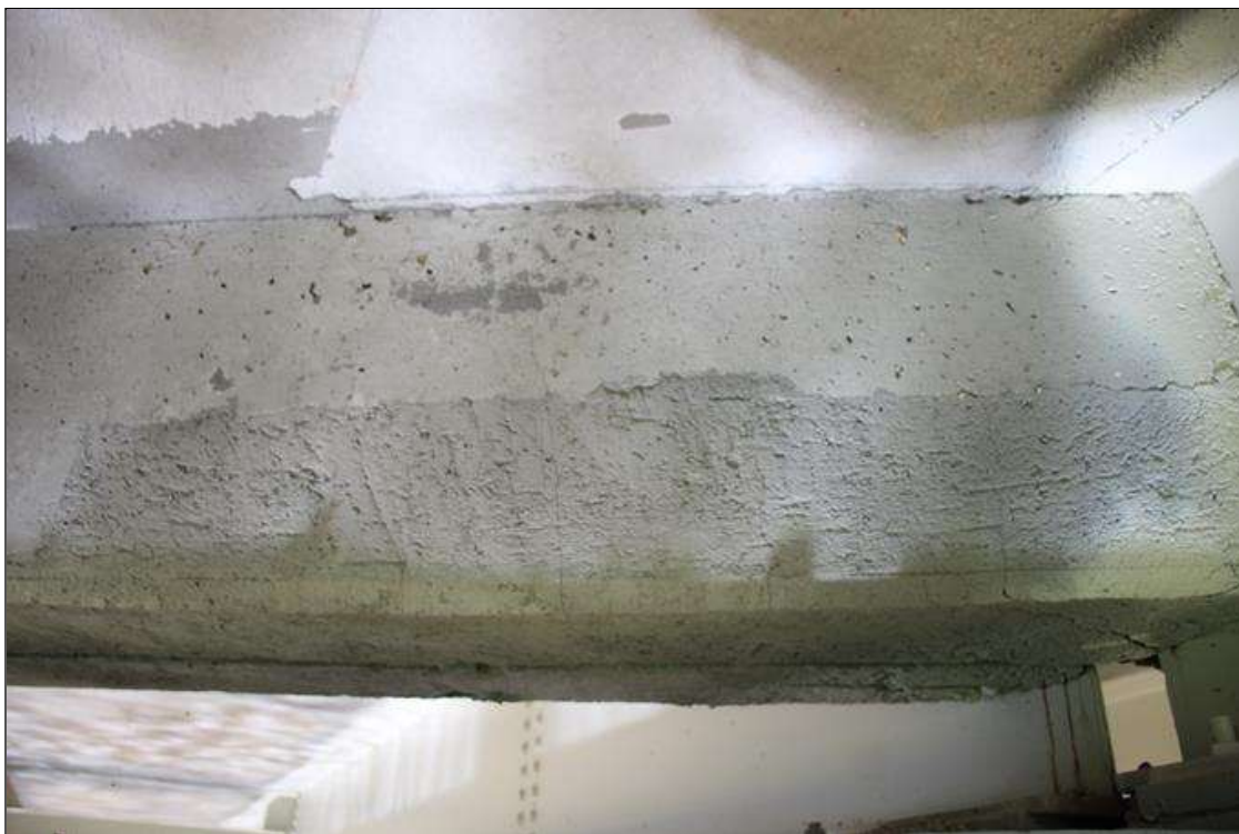
Span 7 Deck: NEW REPAIR: 6 FT LONG X 12 IN HIGH SOUND CONCRETE PATCH BOTTOM OF BAY 3 END DIAPHRAGM, NEXT TO BEAM 3, AT BENT 6. PATCH EXHIBITS UP TO 0.03 IN WIDE VERTICAL CRACKS, SCATTERED.
