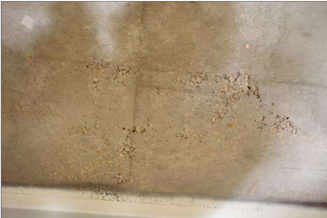
Span 5 Deck: 6 FT LONG X 3 FT WIDE X UP TO 3/4 IN DEEP AREA OF HONEYCOMBING IN BAY 3 NEAR BENT 5.
