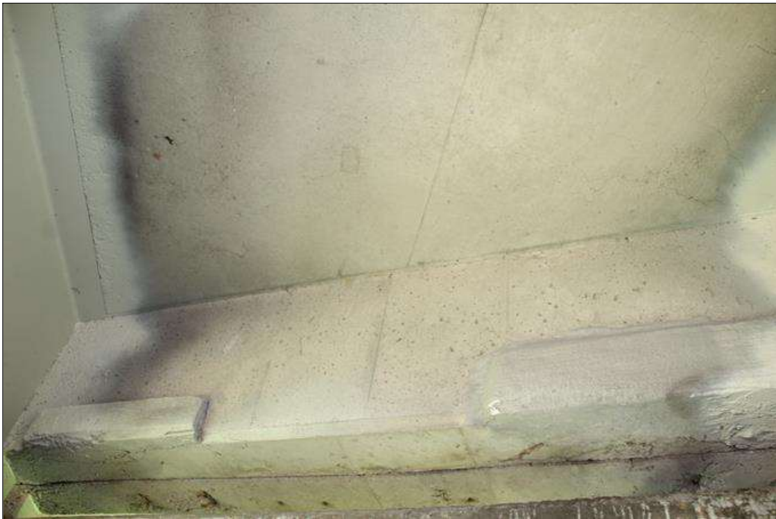
Span 3 Deck: 32 IN LONG X 1 FT HIGH SOUND CONCRETE PATCHES IN PATCHED AREA, BAY 1 END DIAPHRAGM, AT BENT 2.
