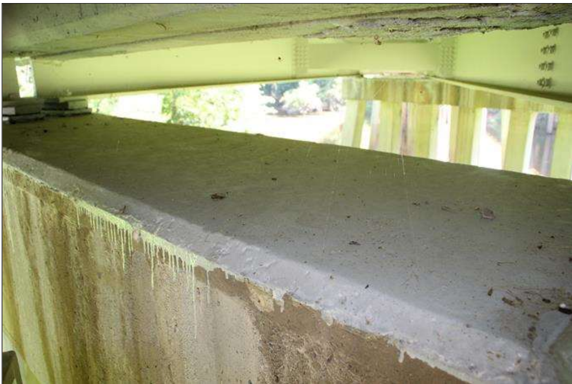
NEW EPOXY SEAL ON TOP OF BENT 1 CAP. TYPICAL ON TOP OF ALL BENTS AND BOTH END BENTS.
