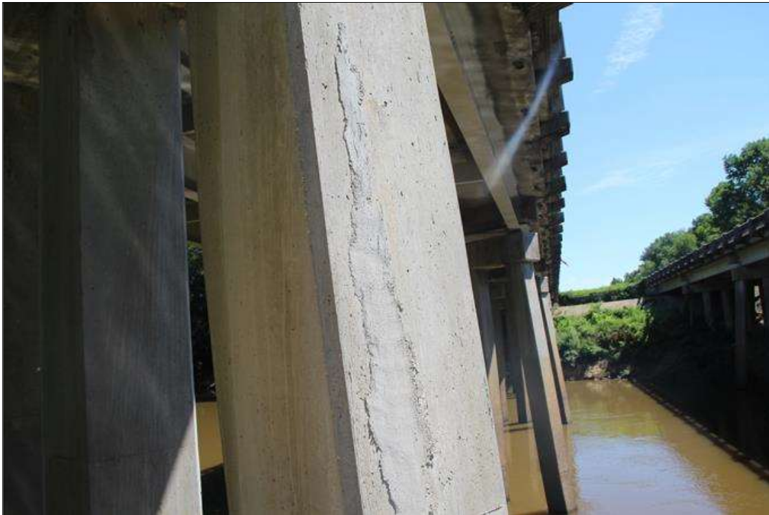
Bent 3 Pile 7: 5 FT HIGH X UP TO 6 IN WIDE CONCRETE PATCH WITH HAIRLINE VERTICAL CRACKS IN EAST FACE, LOCATED AT 4 FT BELOW THE CAP.
