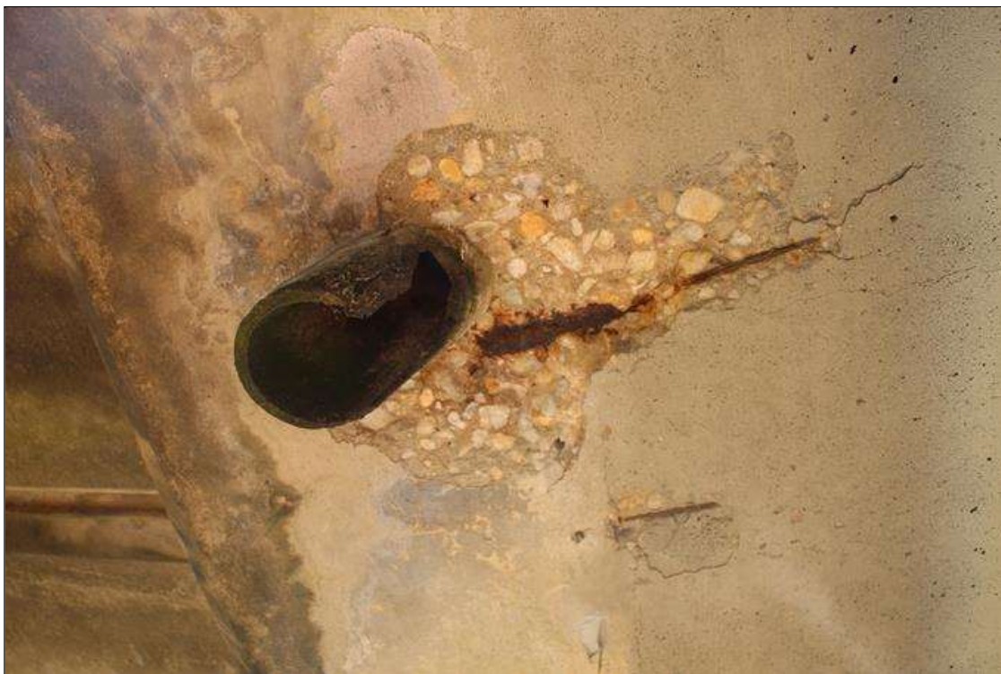
Span 1 Deck: UP TO 1 FT WIDE X 9 IN LONG X UP TO 1 IN DEEP SPALL WITH EXPOSED REINFORCEMENT IN RIGHT OVERHANG, LOCATED AT THIRD DRAIN PIPE. 80% SECTION REMAINING IN EXPOSED REINFORCEMENT.
