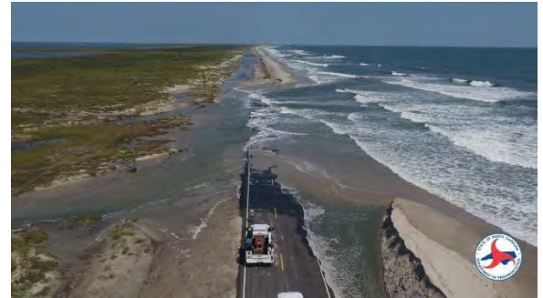
Figure 5J- 5: NC-12 on Ocracoke Island washed out after Hurricane Dorian
