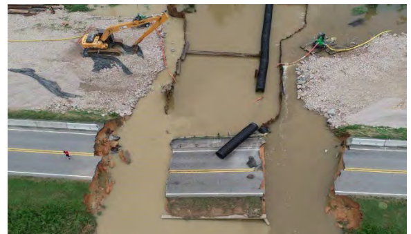
Figure 5J-5: The Little River washed out US- 401 in northeast Wake County
