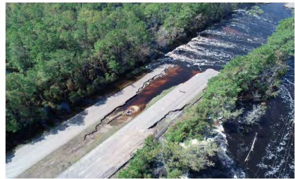
Figure 5J- 2: US-421 at the Pender/New Hanover County Line was closed for 10 days
