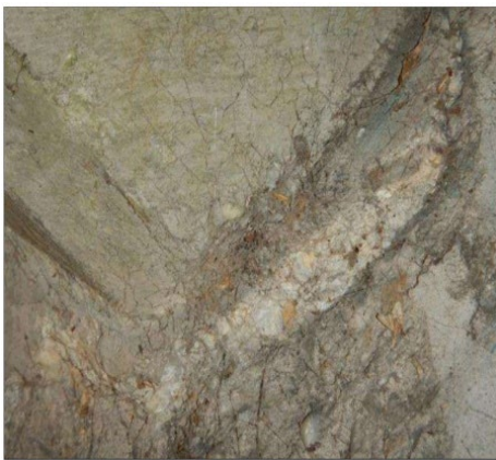
Spall and Delamination
