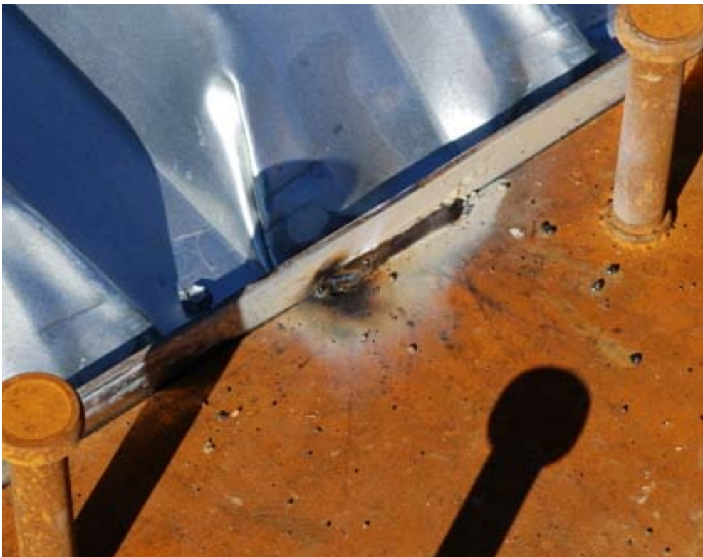
Acceptable weld (slag needs to be removed)
