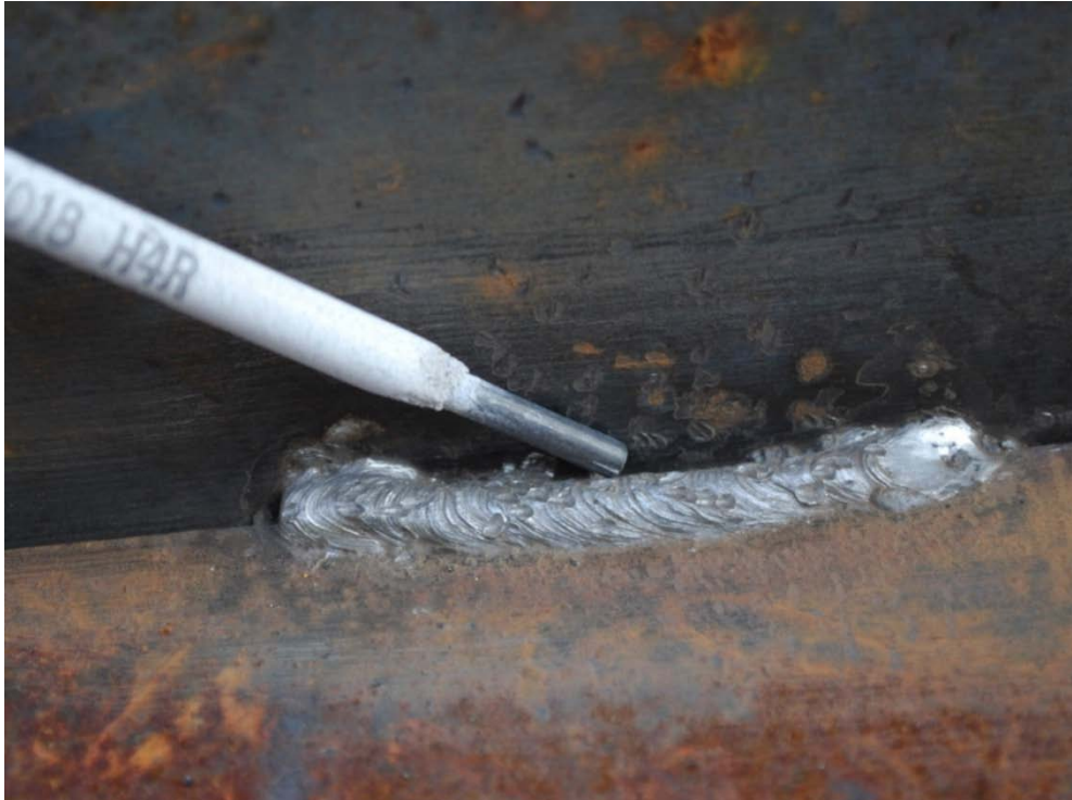
Unacceptable weld (incomplete fusion at the top toe of weld)
