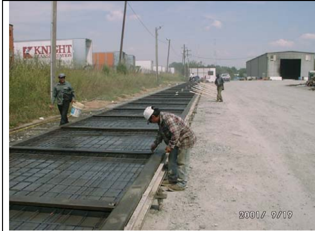
Figure 1: Deck panels being prepared for casting. DURING THE POUR , USE “SPOT CHECK” tabs on the truck chute. AFTER THE POUR , USE “SPOT CHECK” tabs to check the integrity of the components cast. Tabs need to turn BRIGHT PURPLE . For a long square pile, every 15 feet or so.
