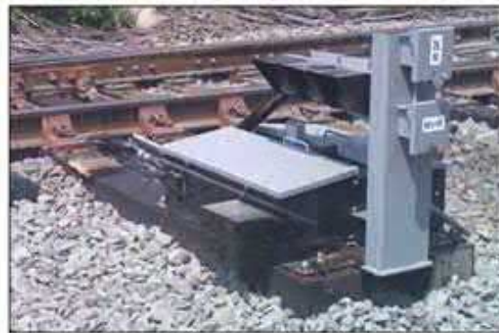
Figure 18: Remote Yard Switch
